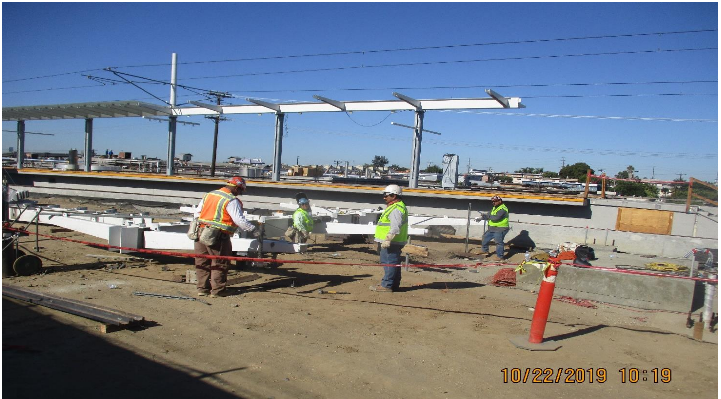
FLORENCE/LA BREA - McMahon Work on ticket plaza canopy at La Brea Station.
