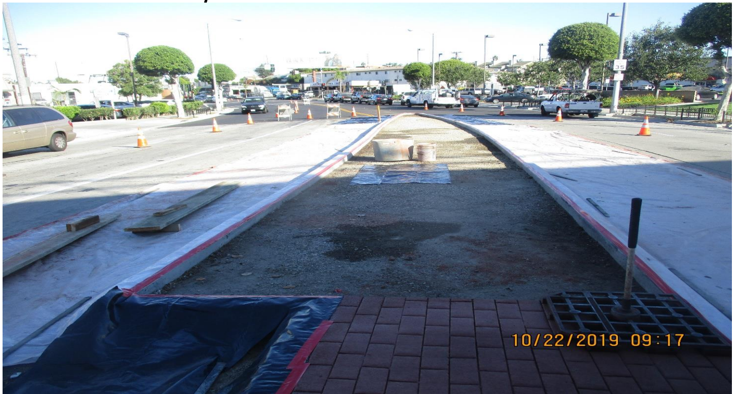
FLORENCE/LA BREA - WSCC Place red stamped concrete at La Brea center island.
