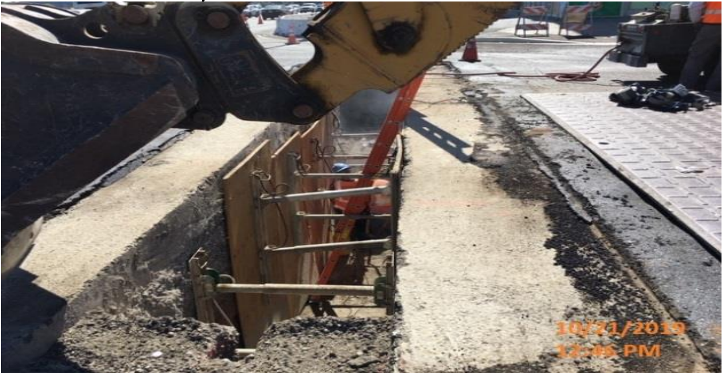
EXPOSITION/CRENSHAW STATION – Continued work on U – Line storm drain on the west side of the intersection of Obama Blvd and Crenshaw Blvd.
