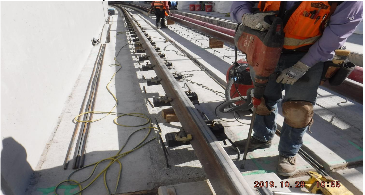
UG3- LKC installation of MPA in the south bond side of UG-3.
