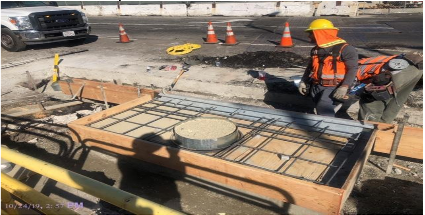
PARK MESA- Manhole collar forming and installing rebar for CB #5 on 60th St & Crenshaw Blvd.
