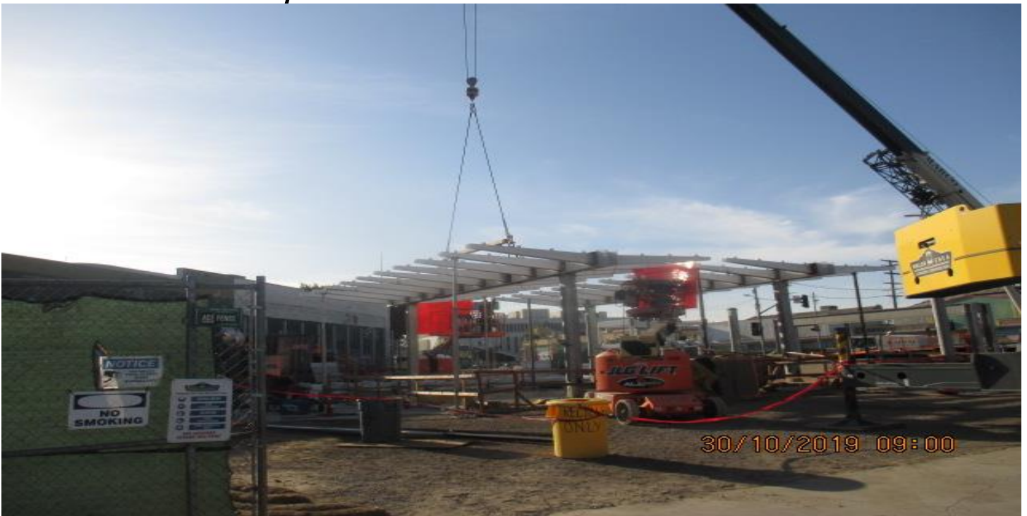
LEIMERT PARK STATION- Setting canopy piece over the main entrance of the portal at the plaza level.
