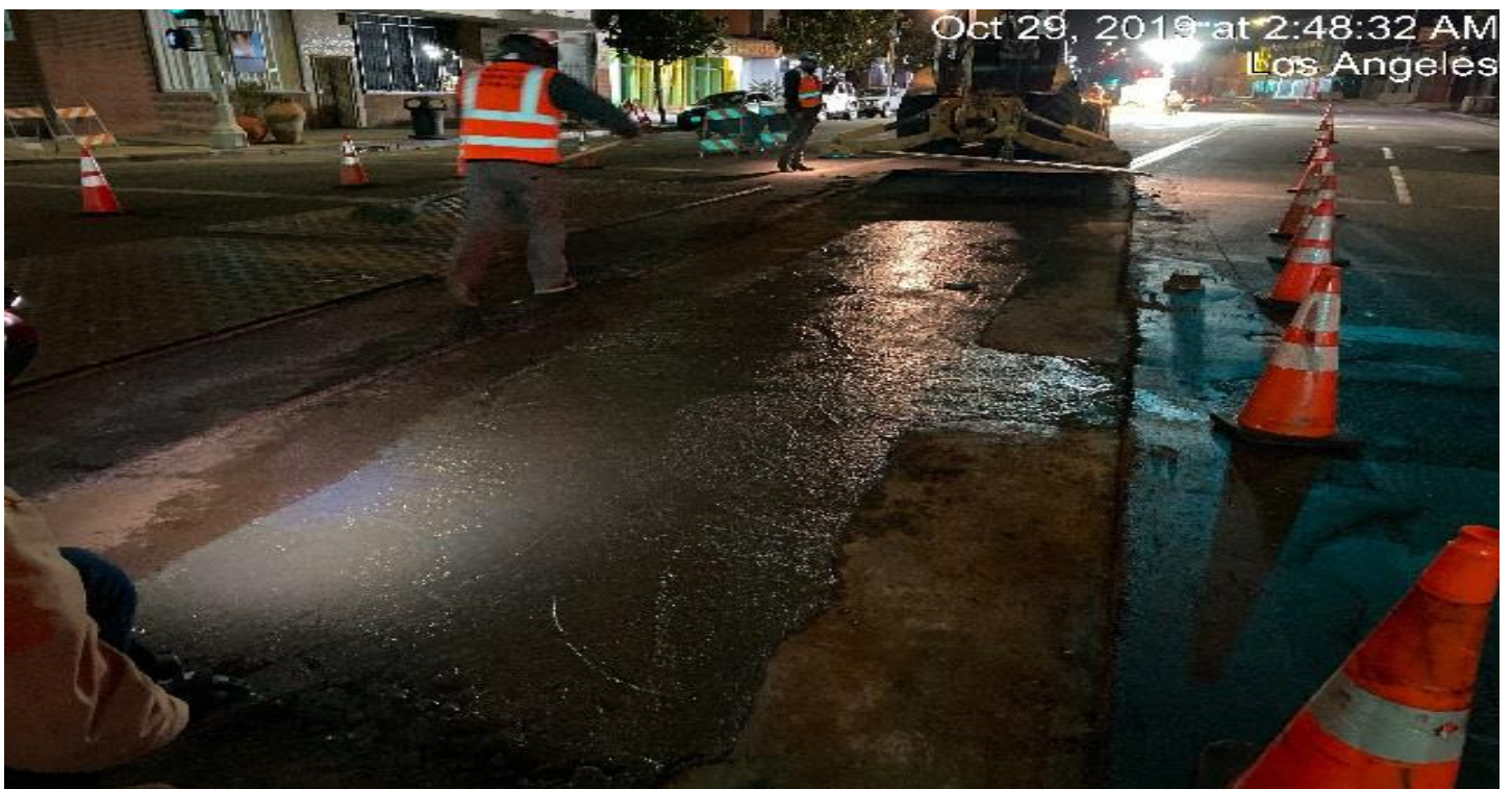
LEIMERT PARK STATION- Placing concrete for PCC roadway on Homeland and Crenshaw Blvd.
