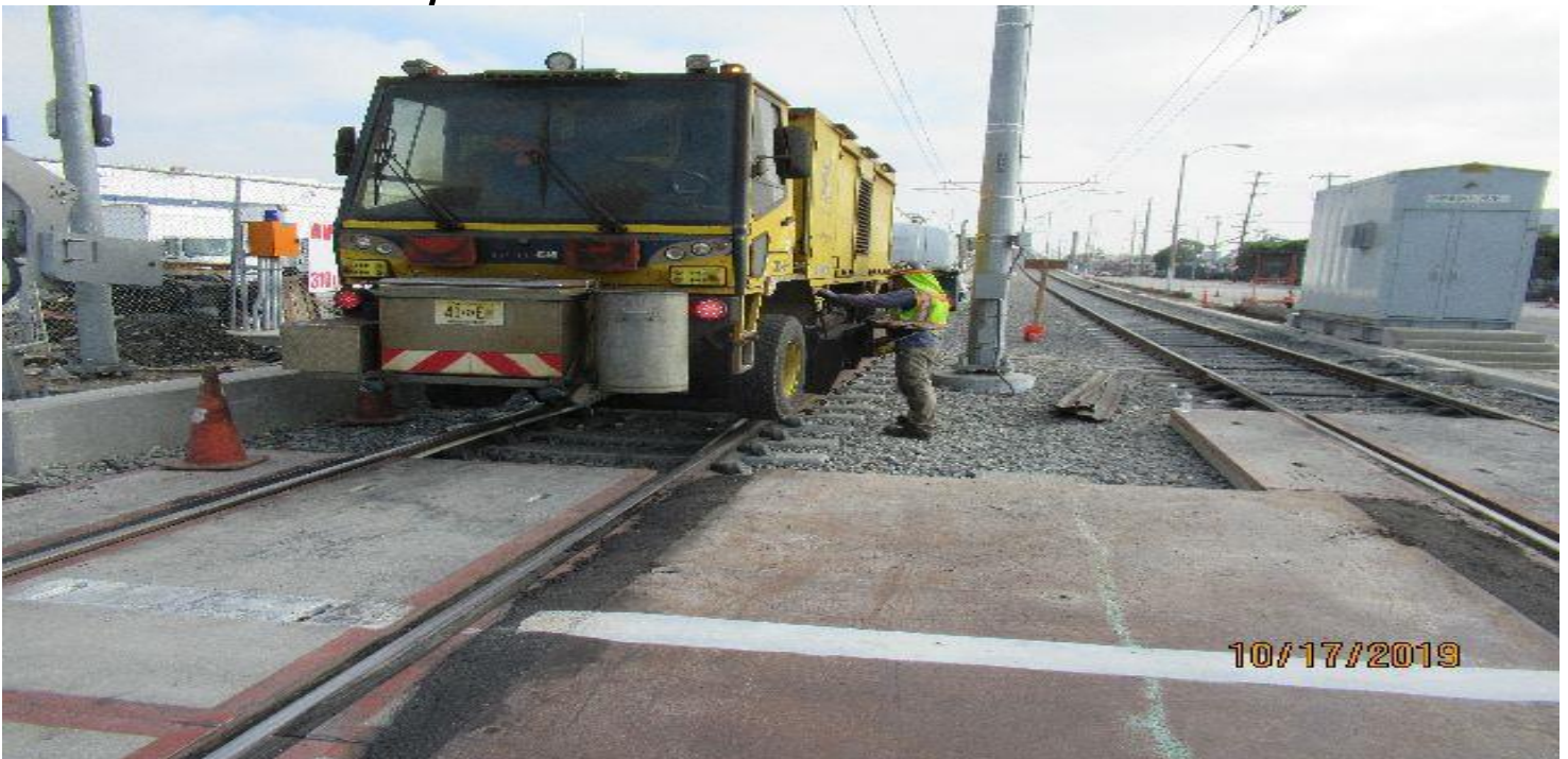
HINDRY AVE – Orgo Therm Weld setting profile work heads to correct profile CPG at Hindry on SB #3 track STA 136+42.
