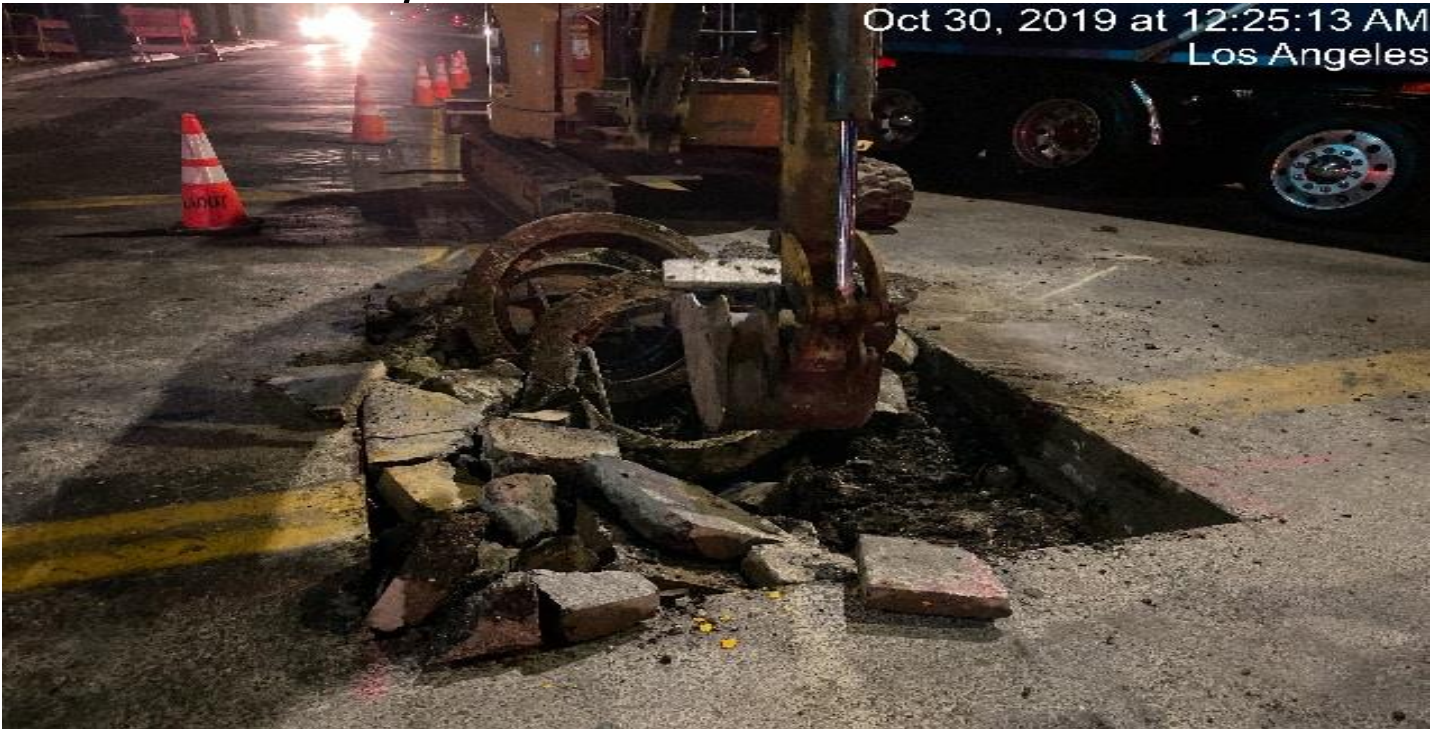
PARK MESA- Excavating to form and cast Manhole #6 on the intersection of 60th St & Crenshaw Blvd.
