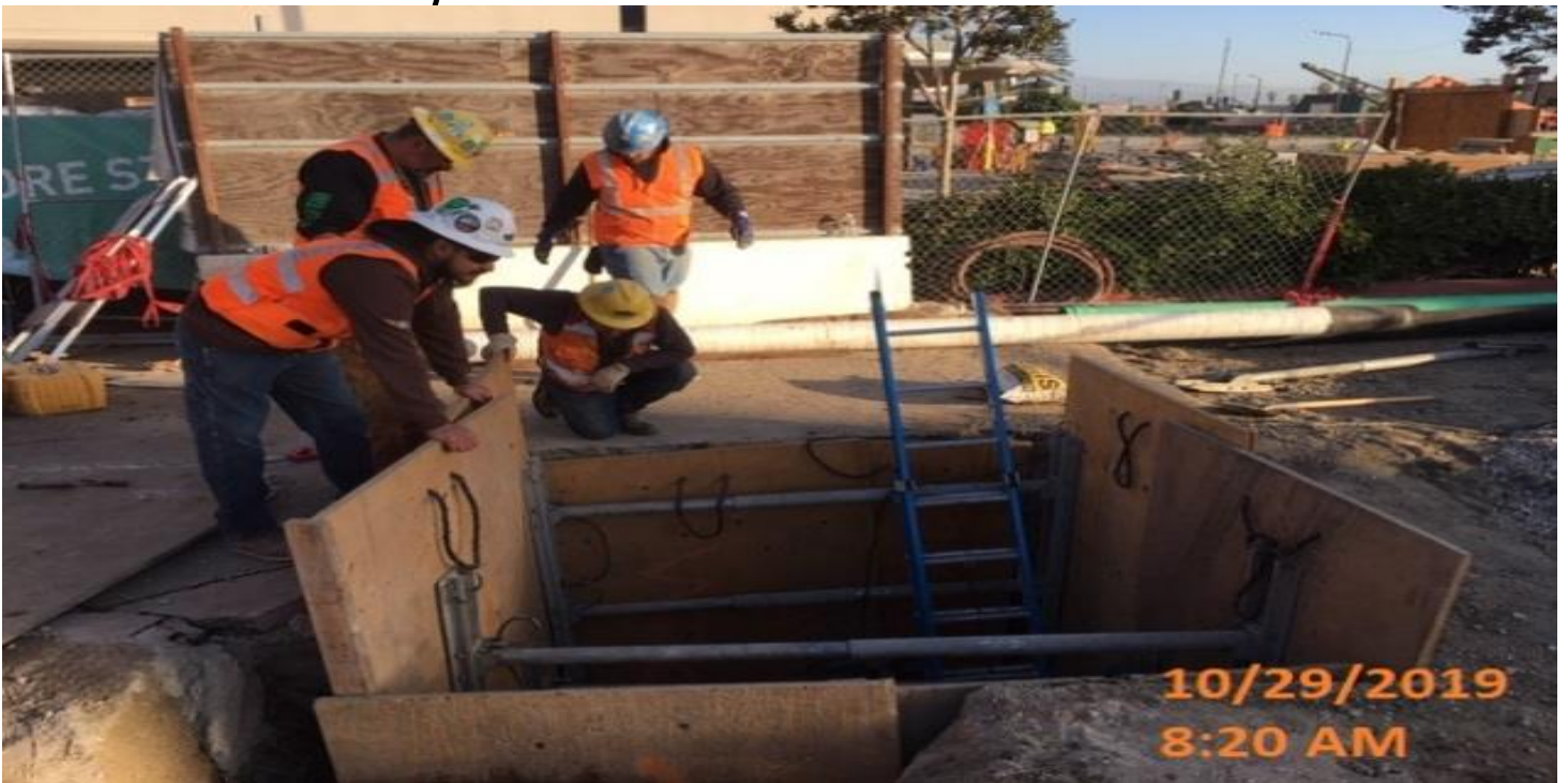
MARTIN LUTHER KING JR. STATION- Forming and excavating Manhole #2 & 3 for Capri E – Line storm drain at the topside.
