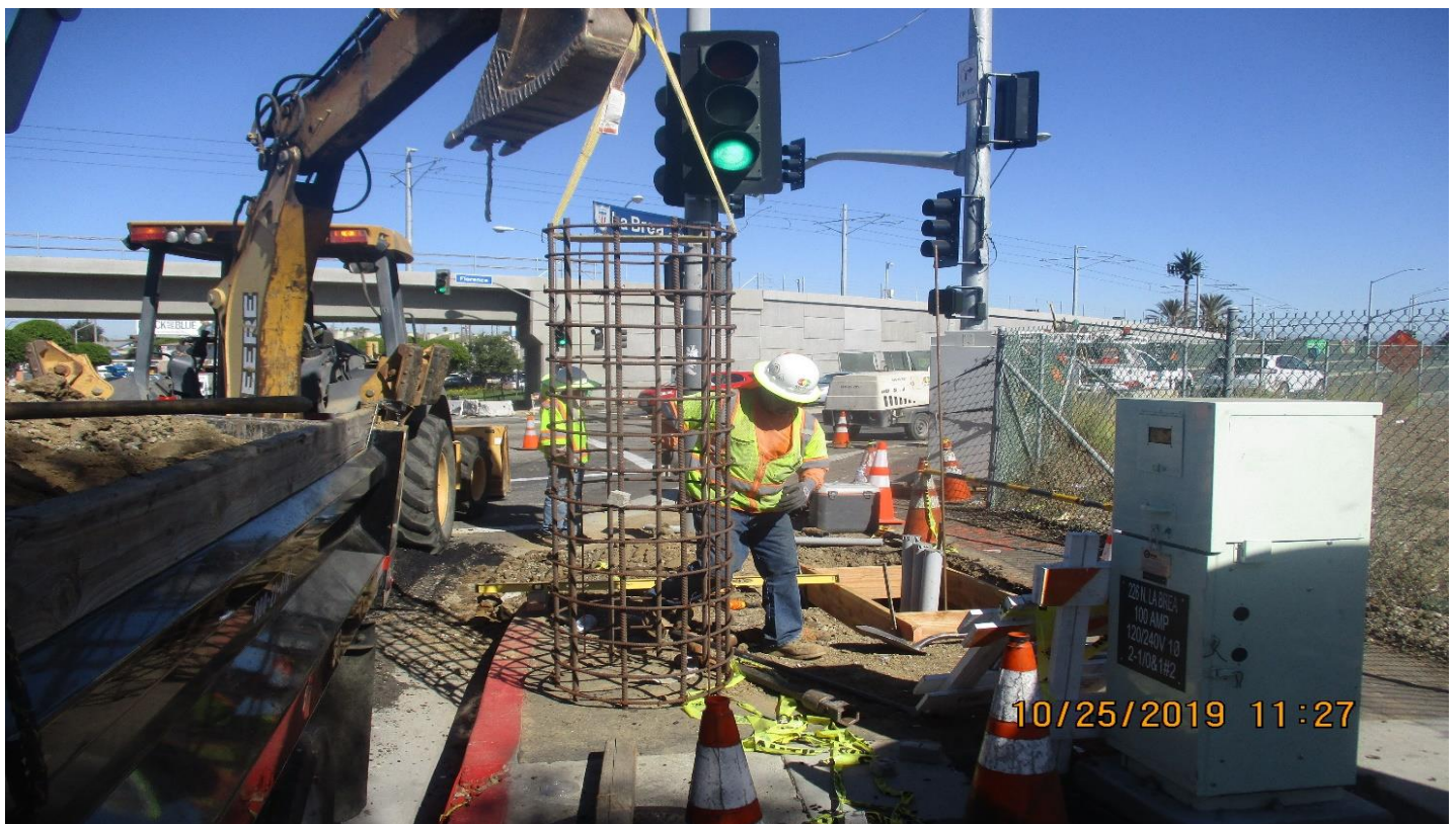
FLORENCE/LA BREA - Select Electric Placed concrete for controller foundation at La Brea.
