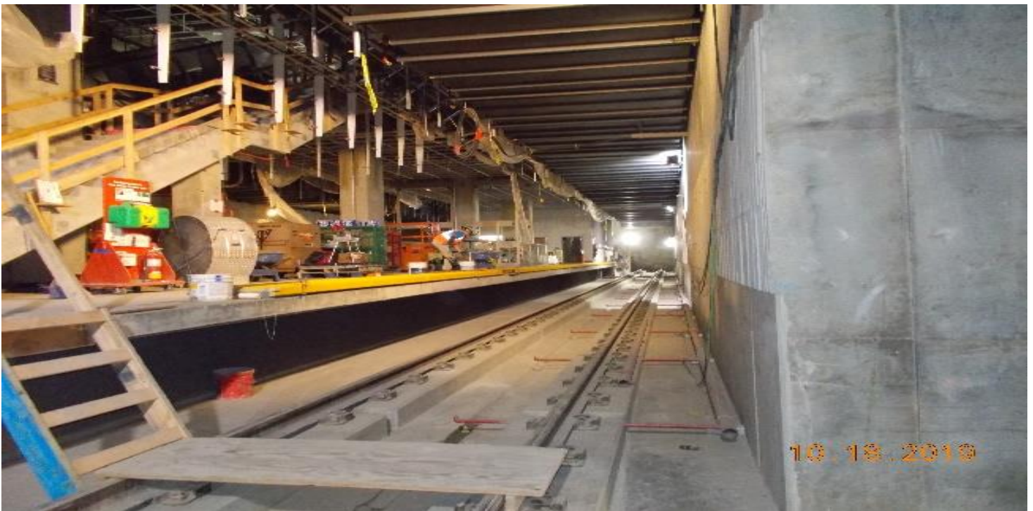
EXPOSITION/CRENSHAW STATION – Continued installation of ADA edge pavers on both sides of the platform level.
