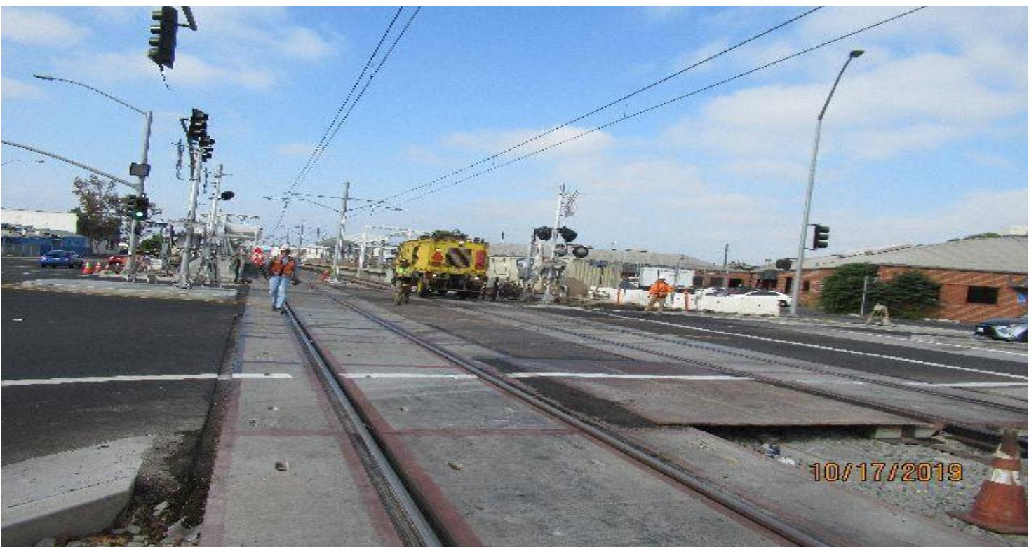
HINDRY AVE – Orgo Therm Weld setting profile grinder onto SB #3 track at Hindry grade crossing.
