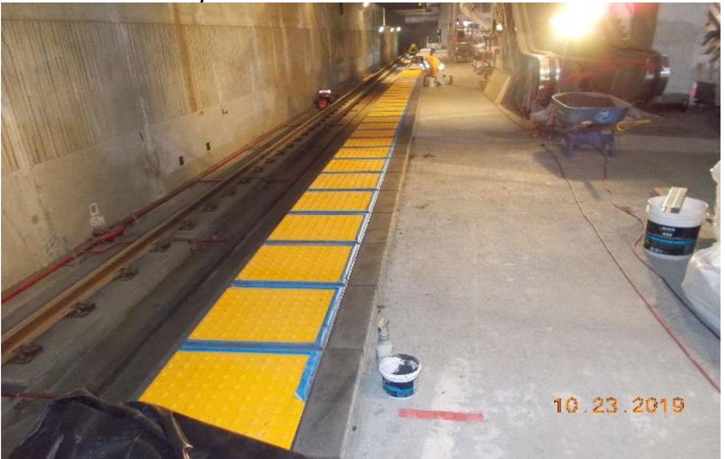
EXPOSITION/CRENSHAW STATION – Continued grouting of ADA edge pavers on both sides of the platform level.
