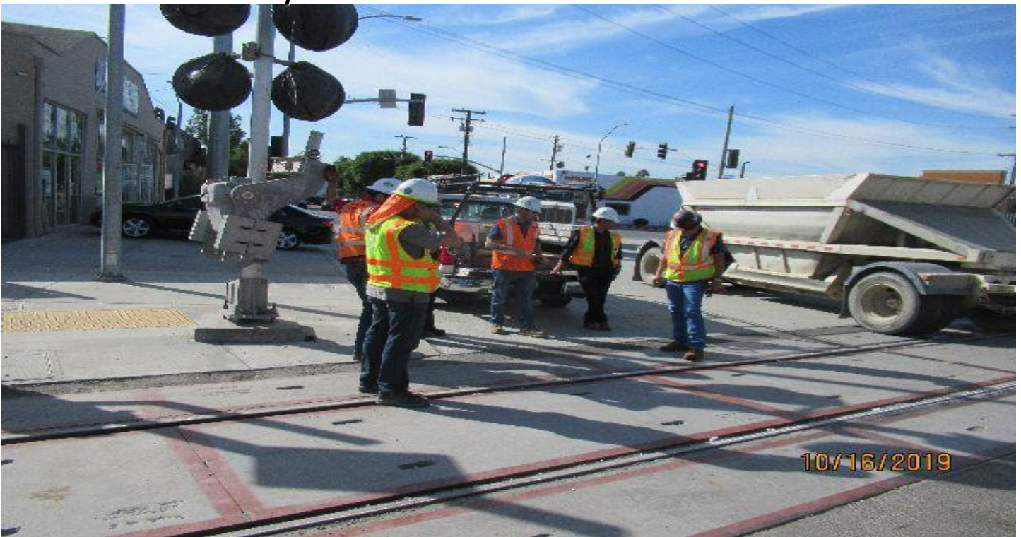
CEDAR AVE – STA 168+46 field walk for rail condition at grade crossings project wide.
