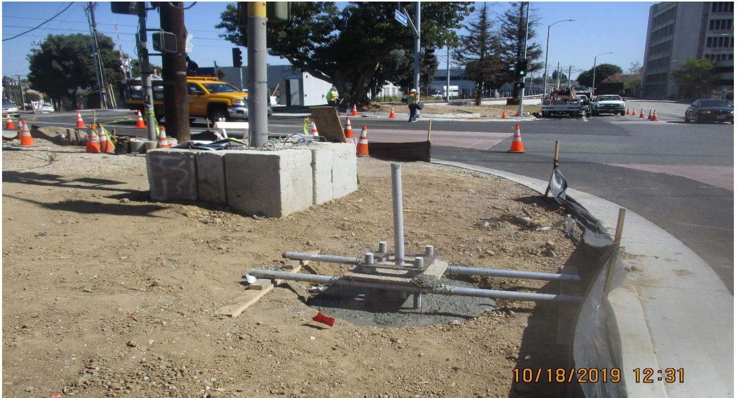
FLORENCE/IVY - Select Electric Placed concrete for TS foundation at Ivy and Florence.
