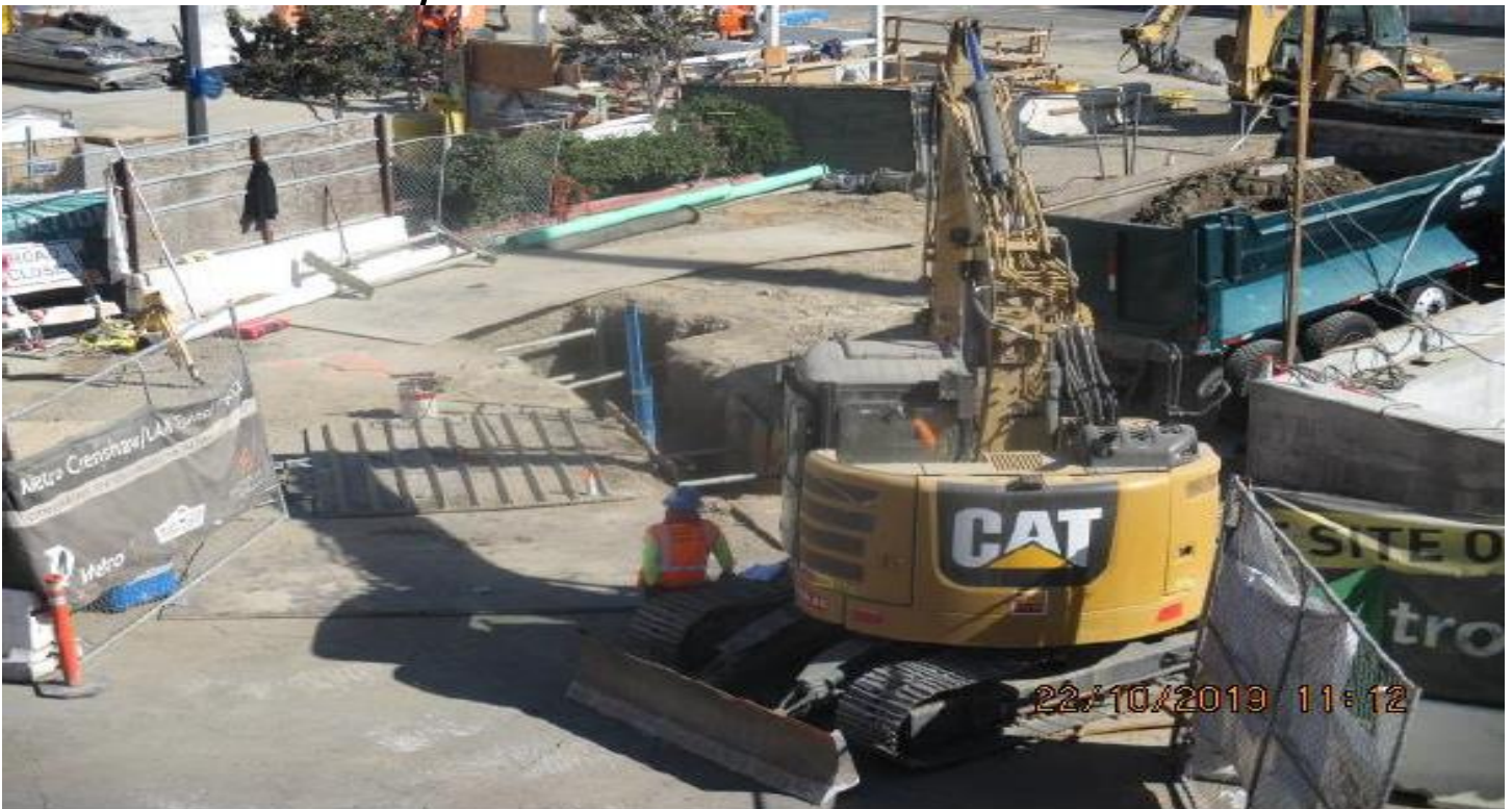
MARTIN LUTHER KING JR. STATION- Excavating Capri sewer line for E – Line storm drain at the topside.
