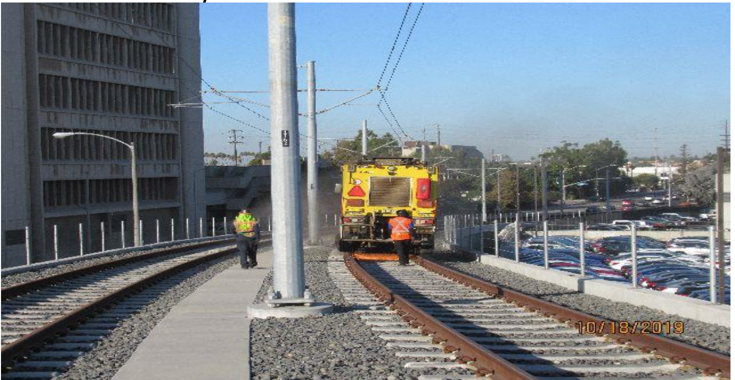
FLORENCE/LA BREA- Orgo Threm Weld Profile grinder on La Brea OP #3 SB track profiling to CPC on both rails threw curves.
