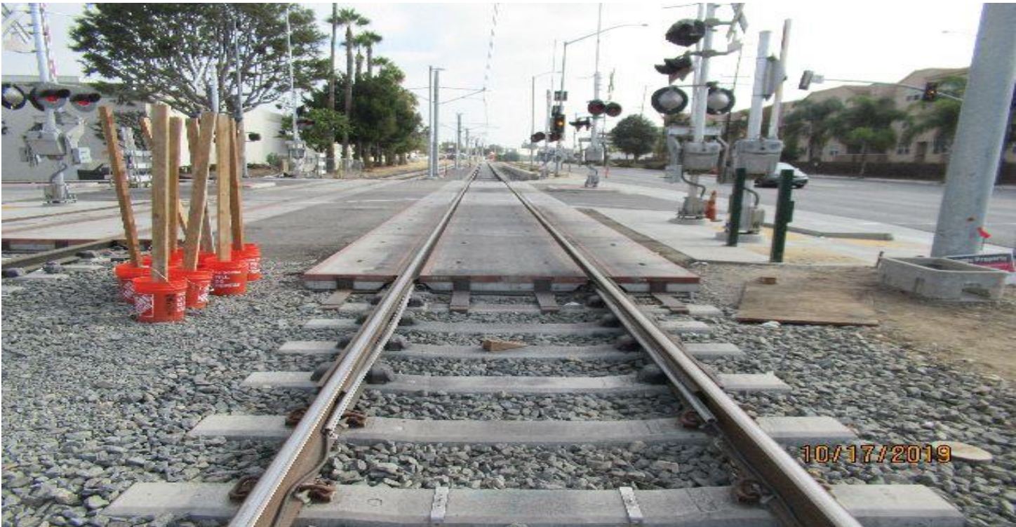
OAK STREET - Oak St. grade crossing NB #4 track final profiling completed STA 136+08.
