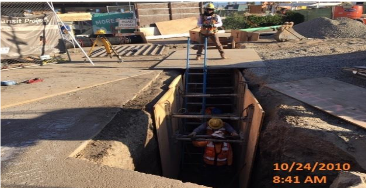
MARTIN LUTHER KING JR. STATION- Installation of Reinforced concrete pipe for Capri E – Line storm drain at the topside.
