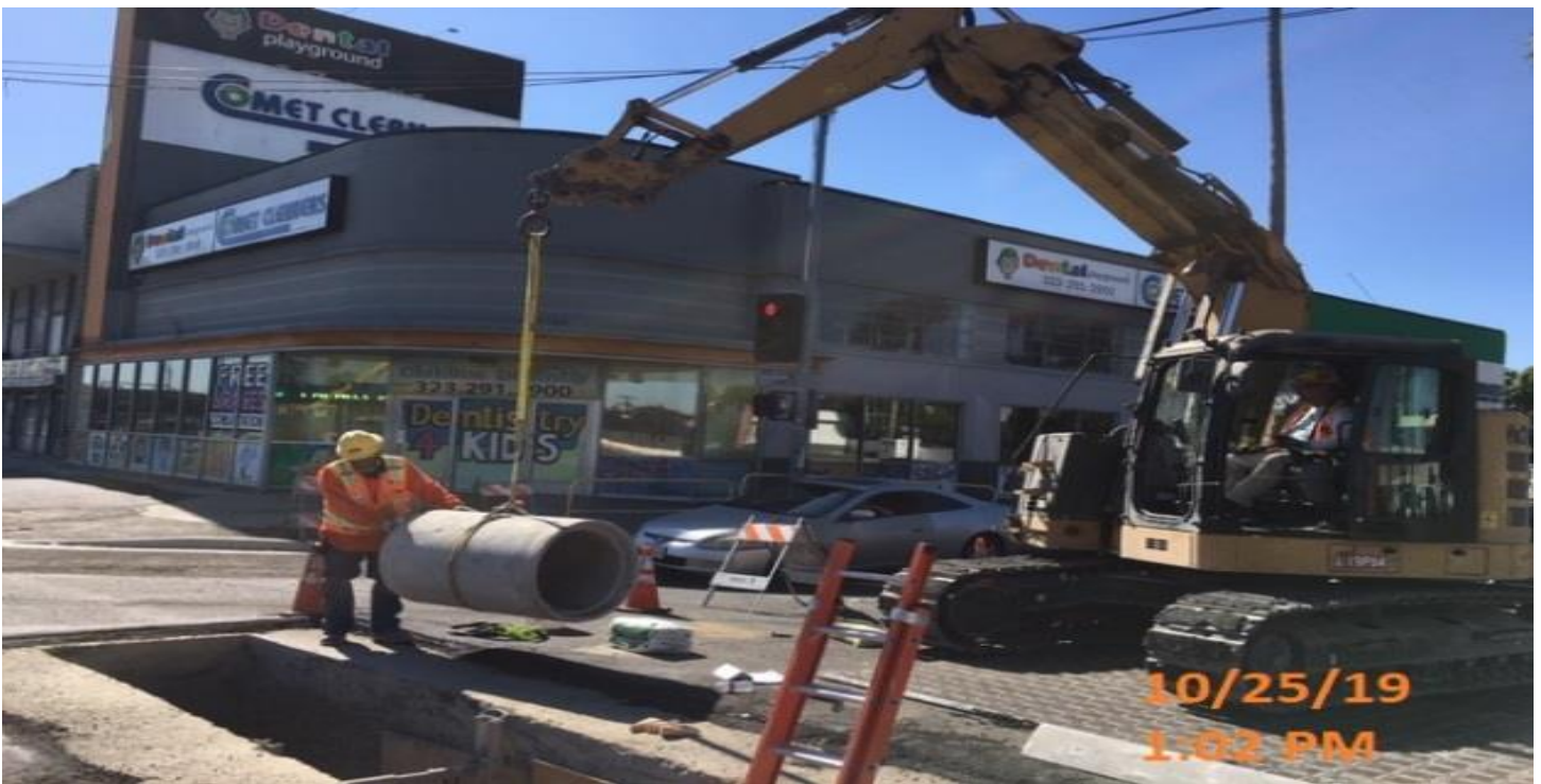
EXPOSITION/CRENSHAW STATION – Placing reinforced concrete pipe for U – Line storm drain on the west side of the intersection of Obama Blvd and Crenshaw Blvd.
