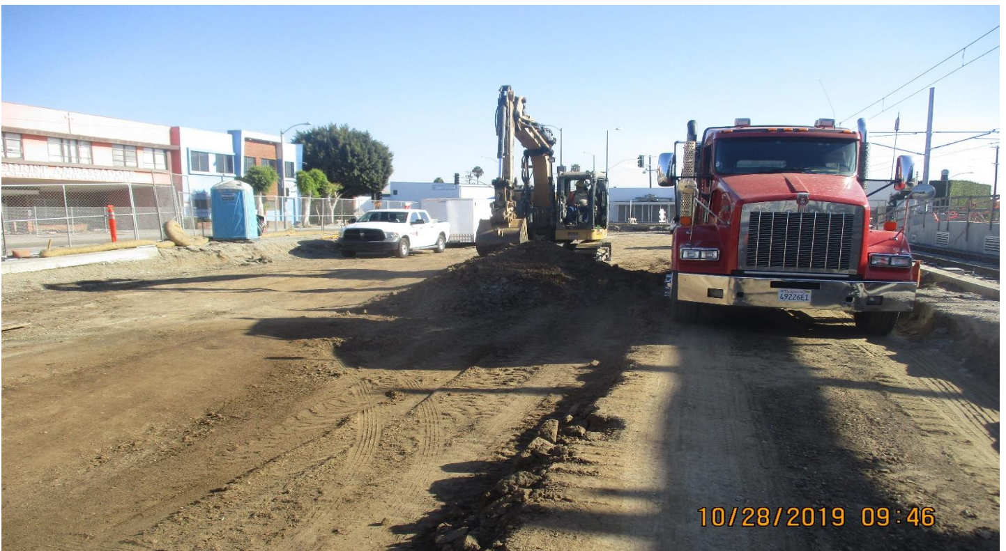
FLORENCE/WEST- WSCC Remove soil and make grade at West Sta parking lot.
