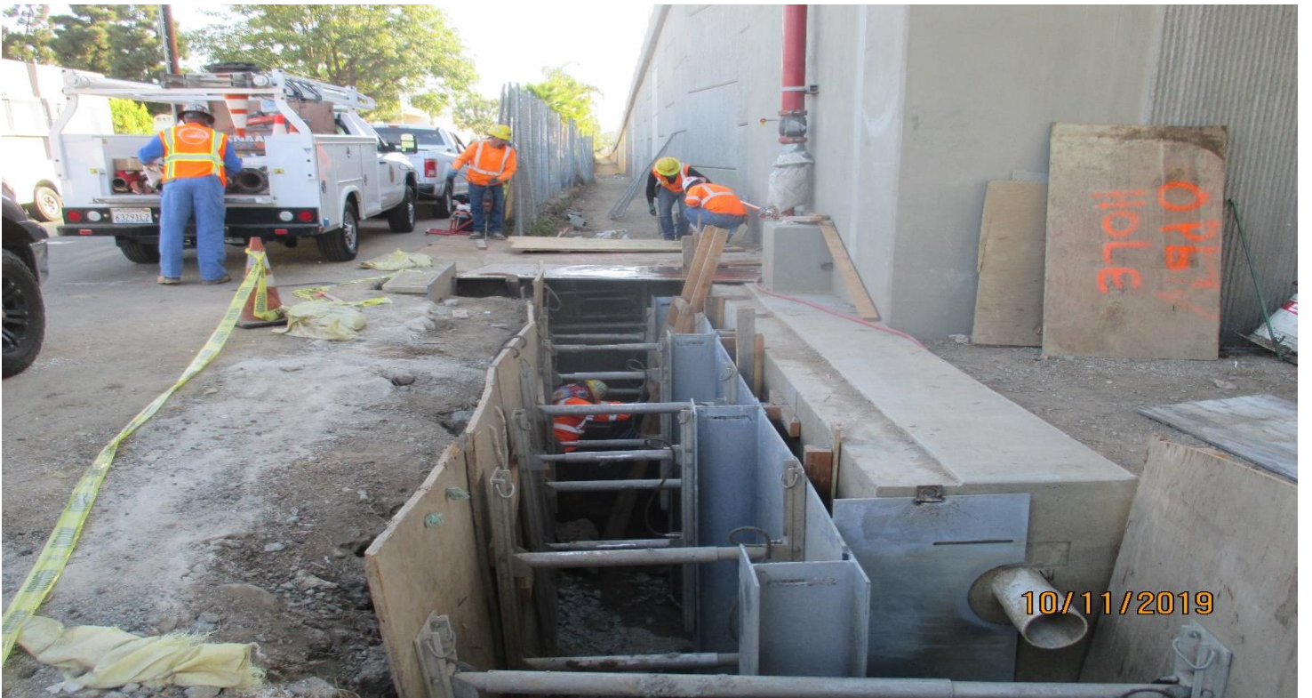
405 BRIDGE - Setting a shoring plate for the COS protection at abutment 5 of the 405
