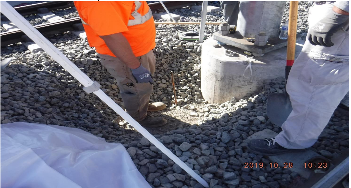
HIGH STREET- STA256+10_lookS_TK ballast disturbance by system work OCR1212 PUNCH LIST.
