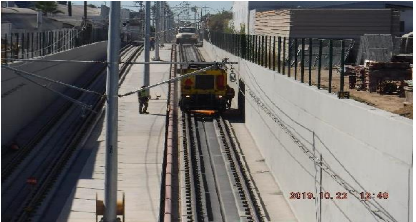
UG3- Rail profiling southbound ramp at Sta 280+00 of the south end portal.
