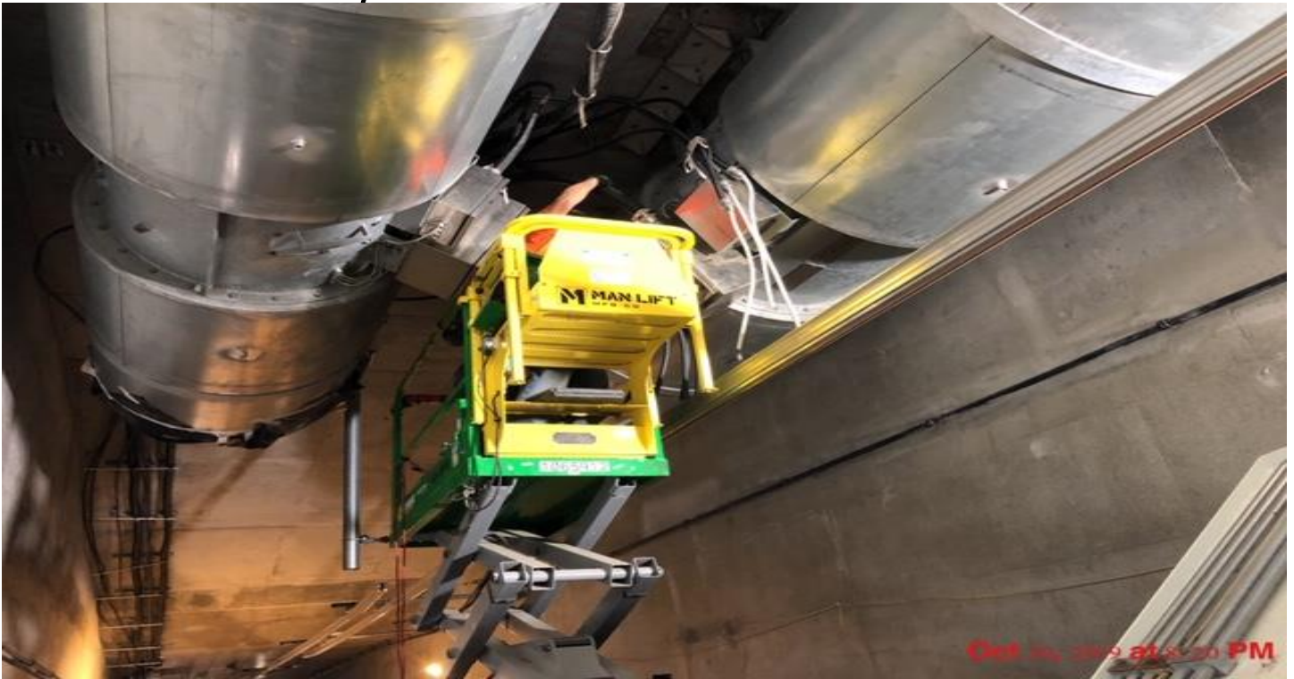
UG3- Continued connecting fire rated cables for the tunnel booster fans on the northbound tunnel at Sta 307+42.
