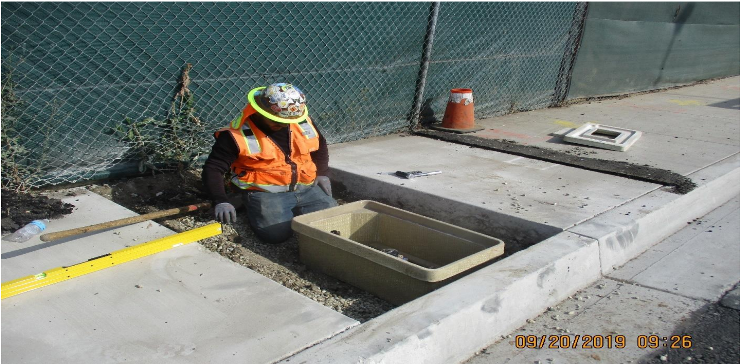
FLORENCE/LA BREA- Bali Construction Place meter boxes and AC back fill water line trenches to La Brea Station.
