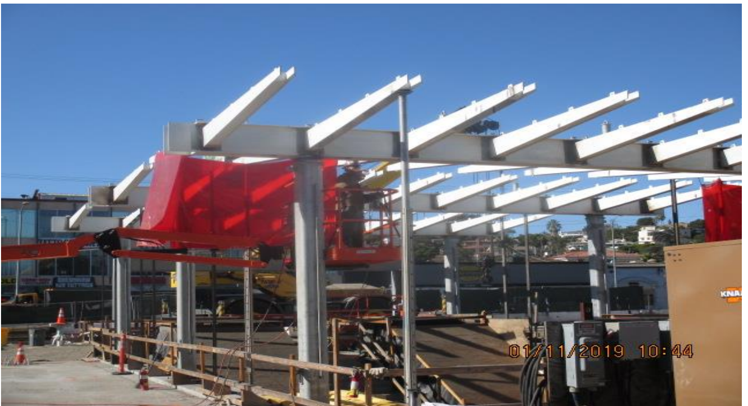
LEIMERT PARK STATION- Continued welding main beam connection for main entrance canopy portal at the plaza level.
