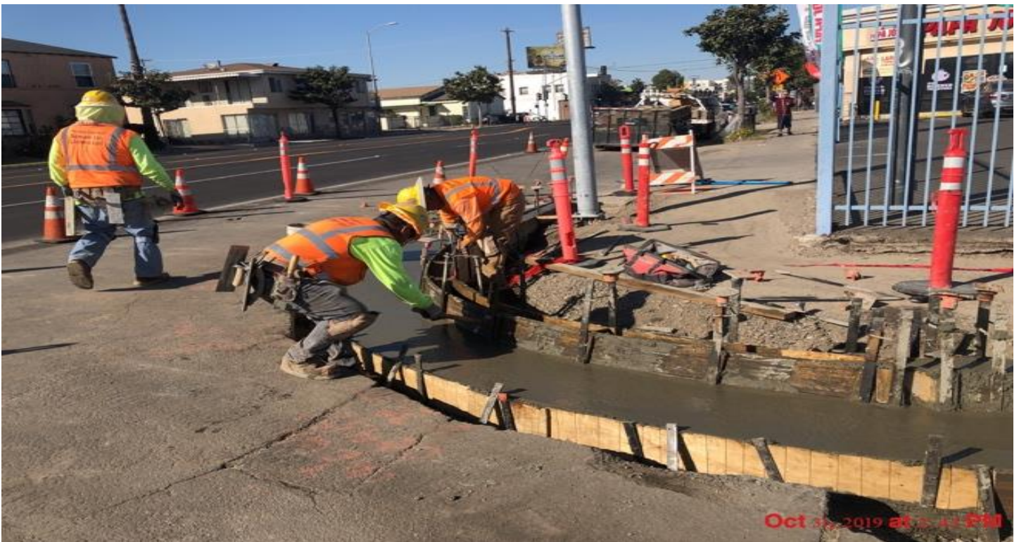
PARK MESA- Curb and gutter placement on the northeast corner of 66th St & Crenshaw Blvd.
