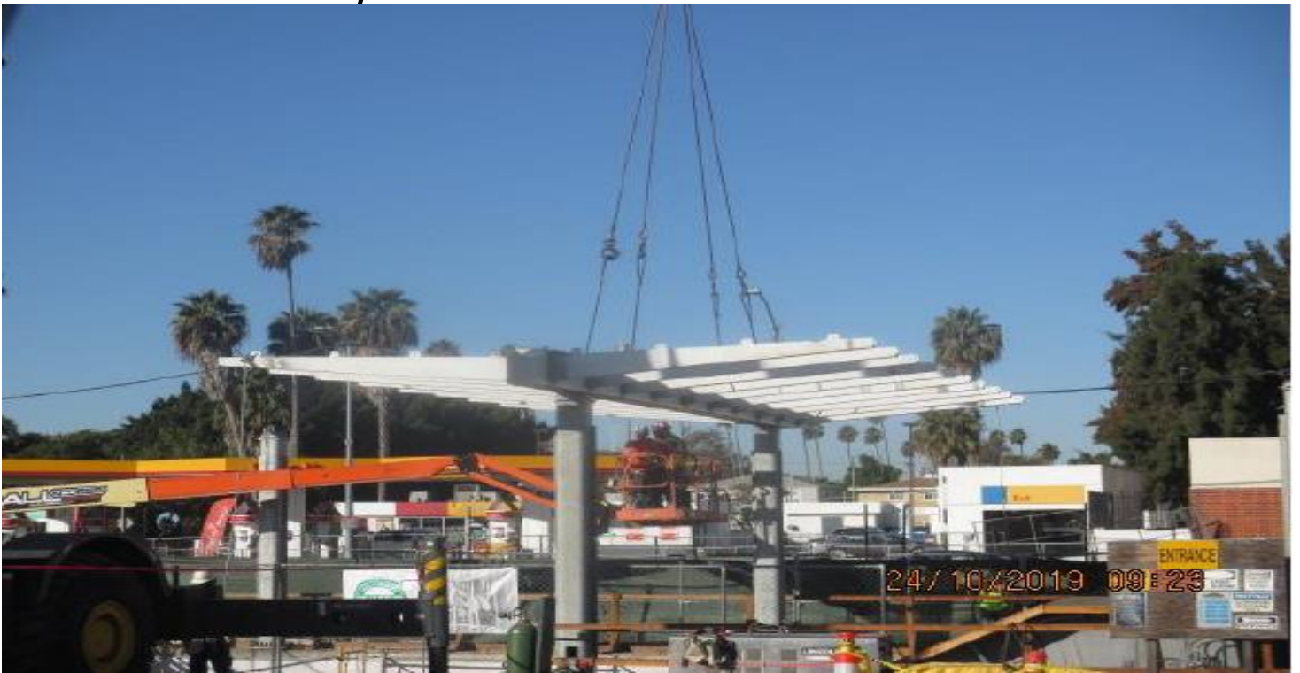
EXPOSITION/CRENSHAW STATION – Setting center canopy piece over the main entrance of the portal at the plaza level.
