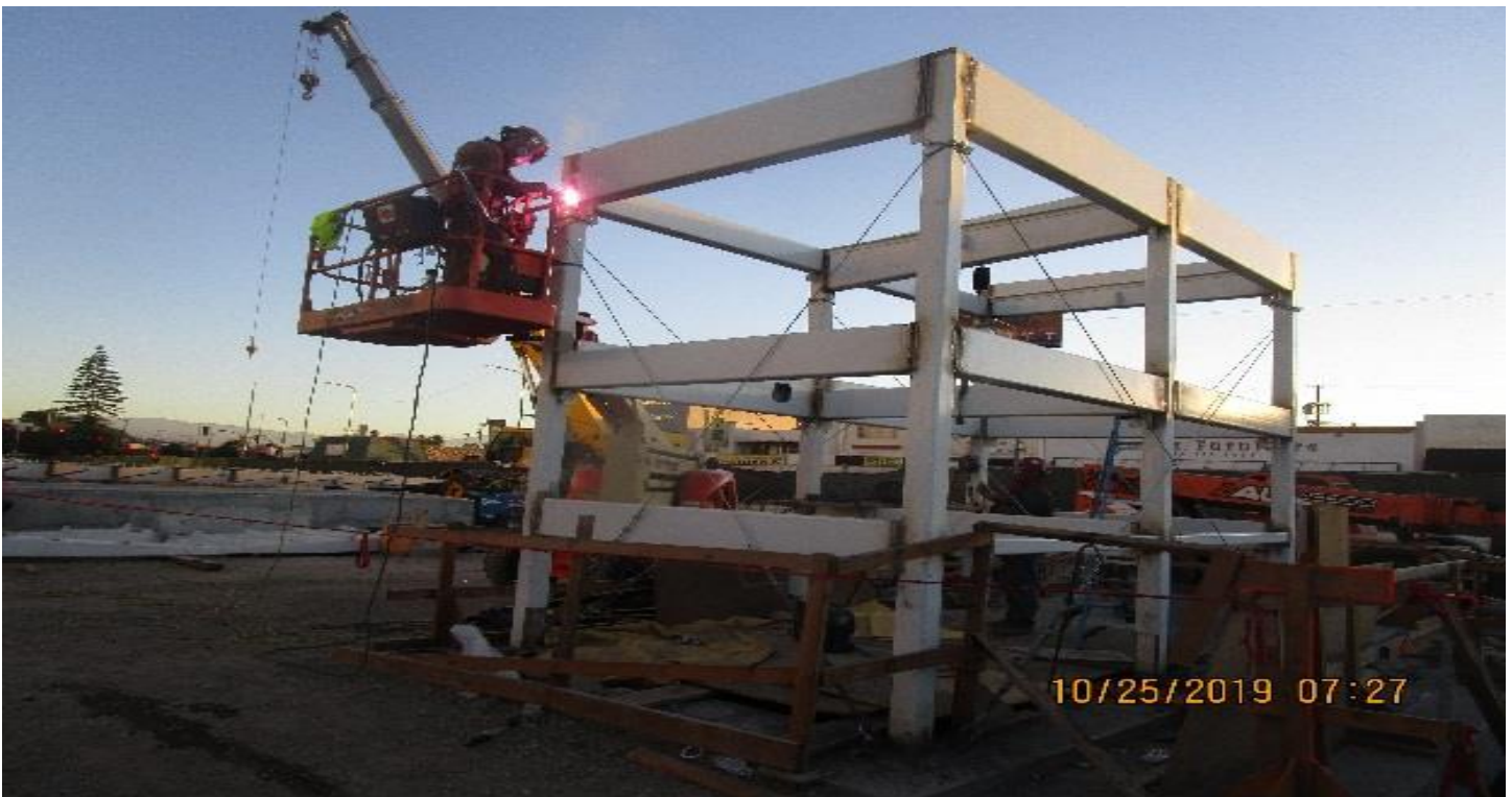
MARTIN LUTHER KING JR. STATION- Continued welding column beam connections for Elevator 1 & 2 at the plaza level.
