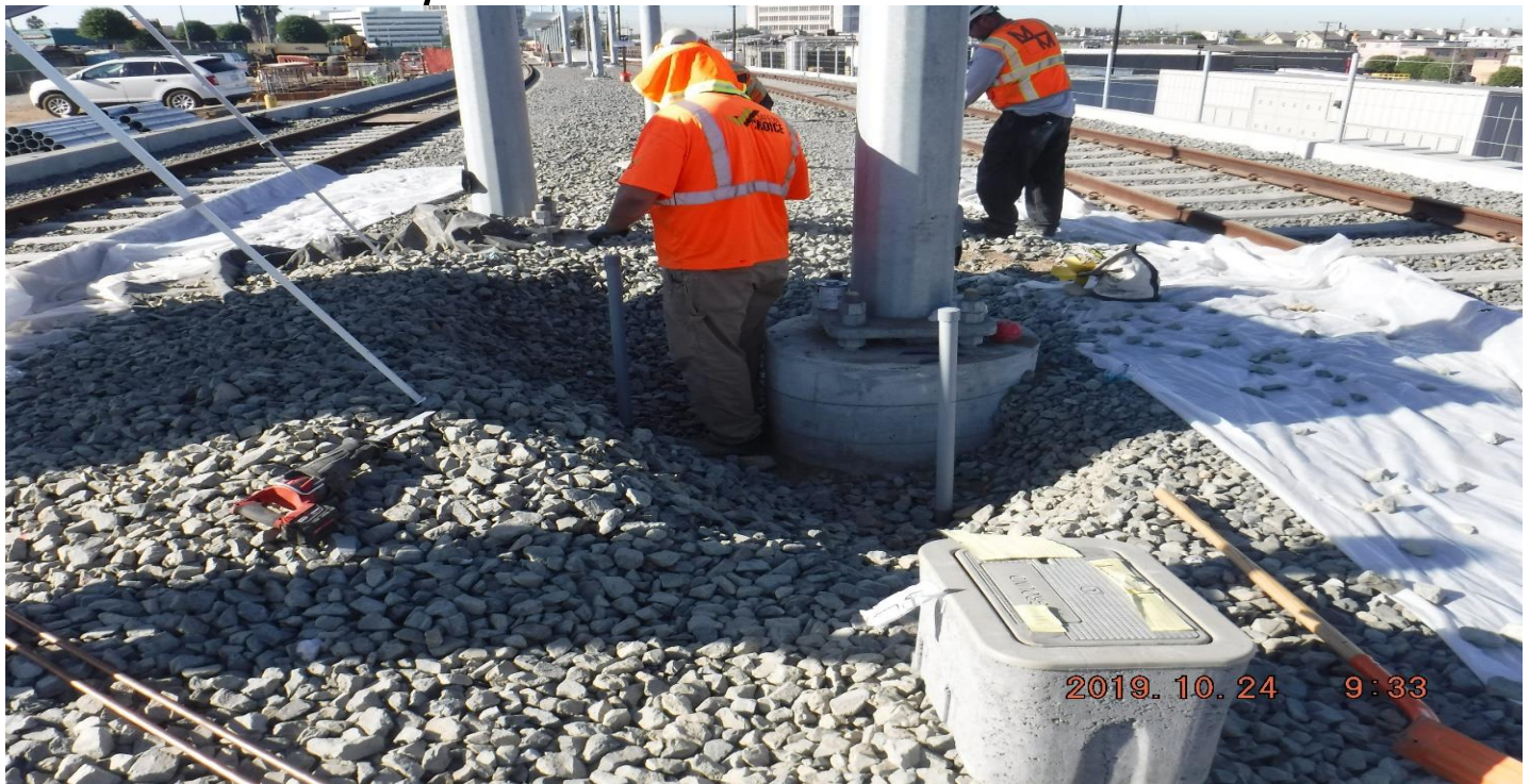
FLORENCE/LA BREA - STA214+00_ Looking South_ TK ballast re-disturbance by system work_OCR1177S_PUNCH LIST.
