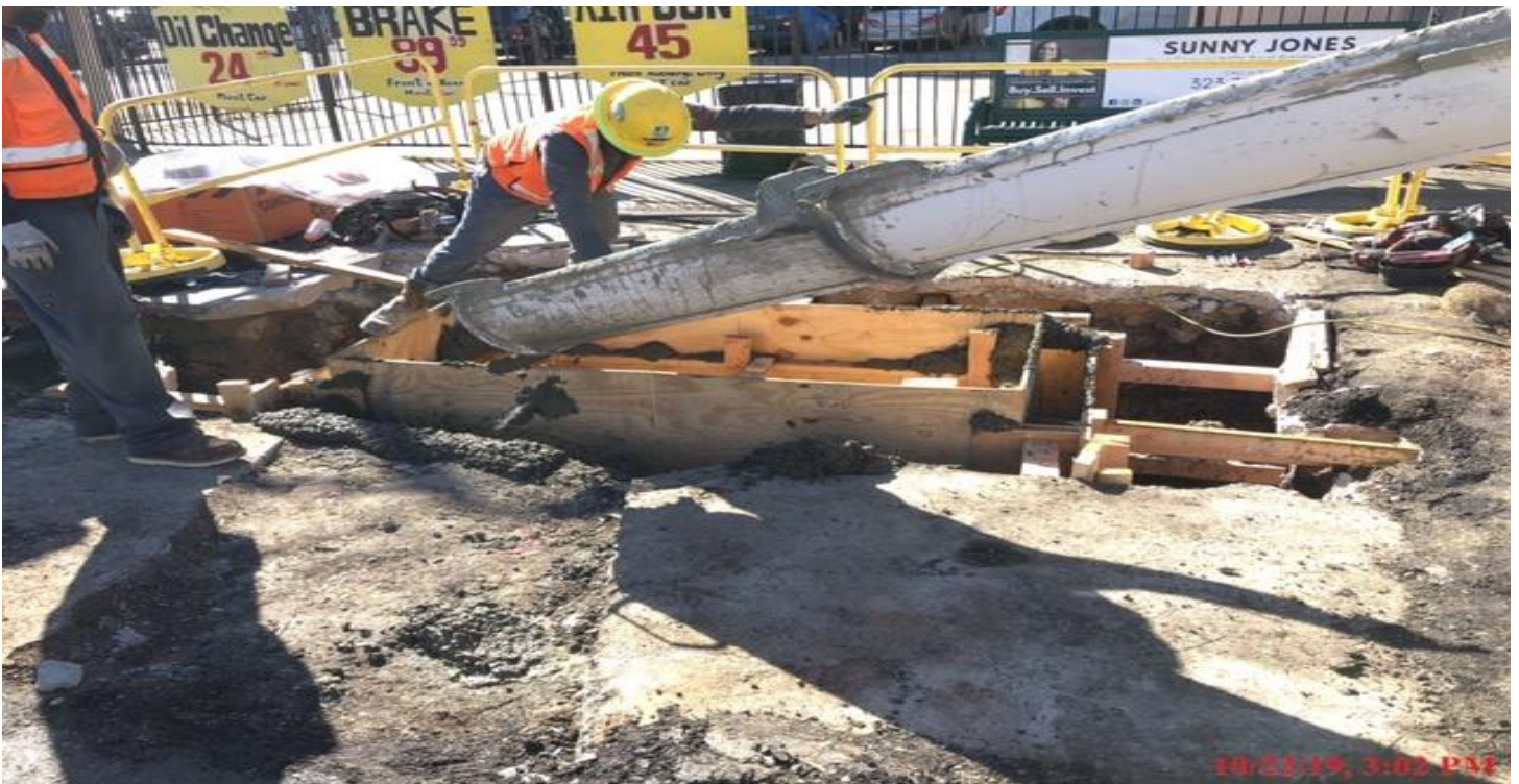
PARK MESA- Placing case 5 encasement for Catch Basin #5 on 60th St & Crenshaw Blvd.
