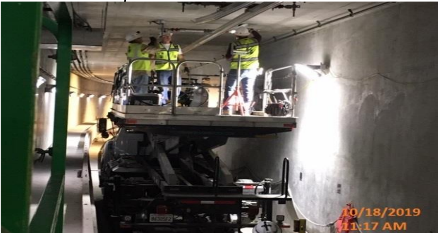
UG3- Continued installation of overhead conductor rail for contact system on the southbound tunnel at Sta 286+56.
