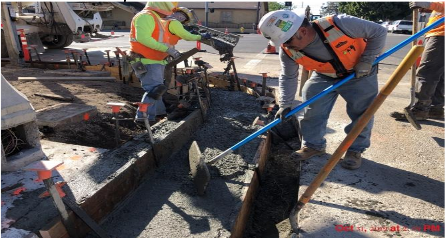
PARK MESA- Curb and gutter placement on the southeast corner of 63rd St & Crenshaw Blvd.
