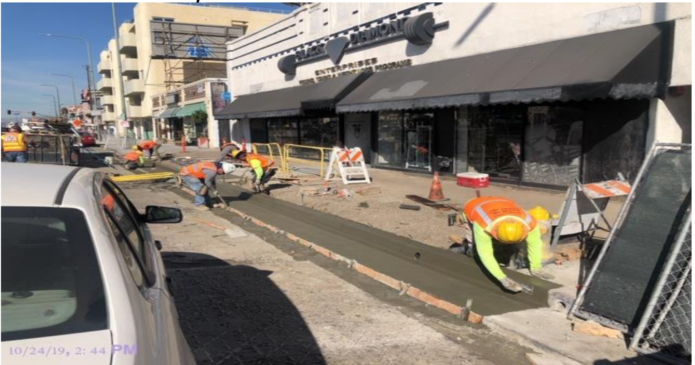
PARK MESA- Continued curb and gutter placement on the northbound side of Crenshaw Blvd from 54th to 57th St.
