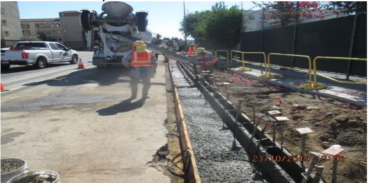
PARK MESA- Curb and gutter placement on the southbound side of 60th St & Crenshaw Blvd.
