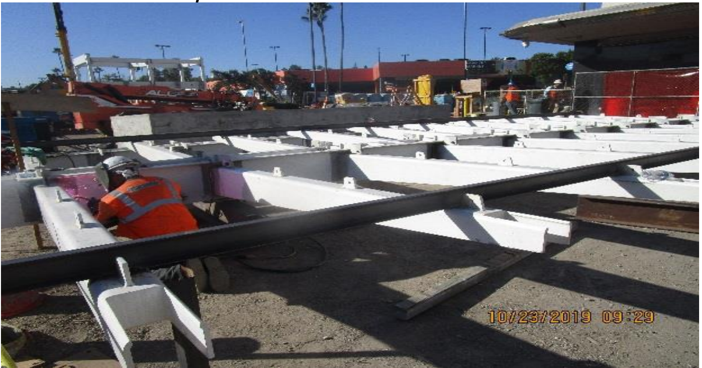
MARTIN LUTHER KING JR. STATION- Continued welding outriggers to main beam connection for main entrance canopy portal.
