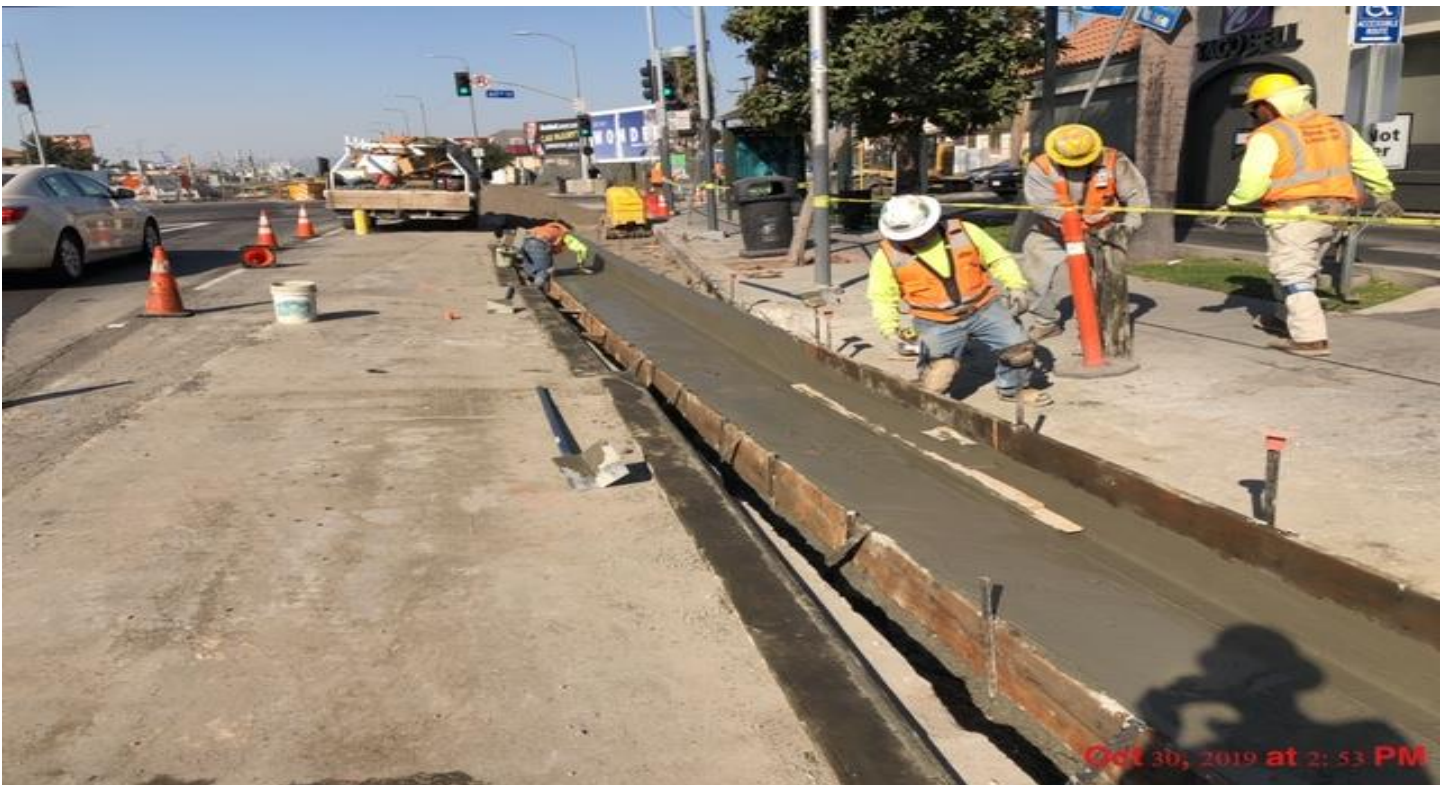
PARK MESA- Curb and gutter placement for bus pad on the southeast corner of 60th St & Crenshaw Blvd.
