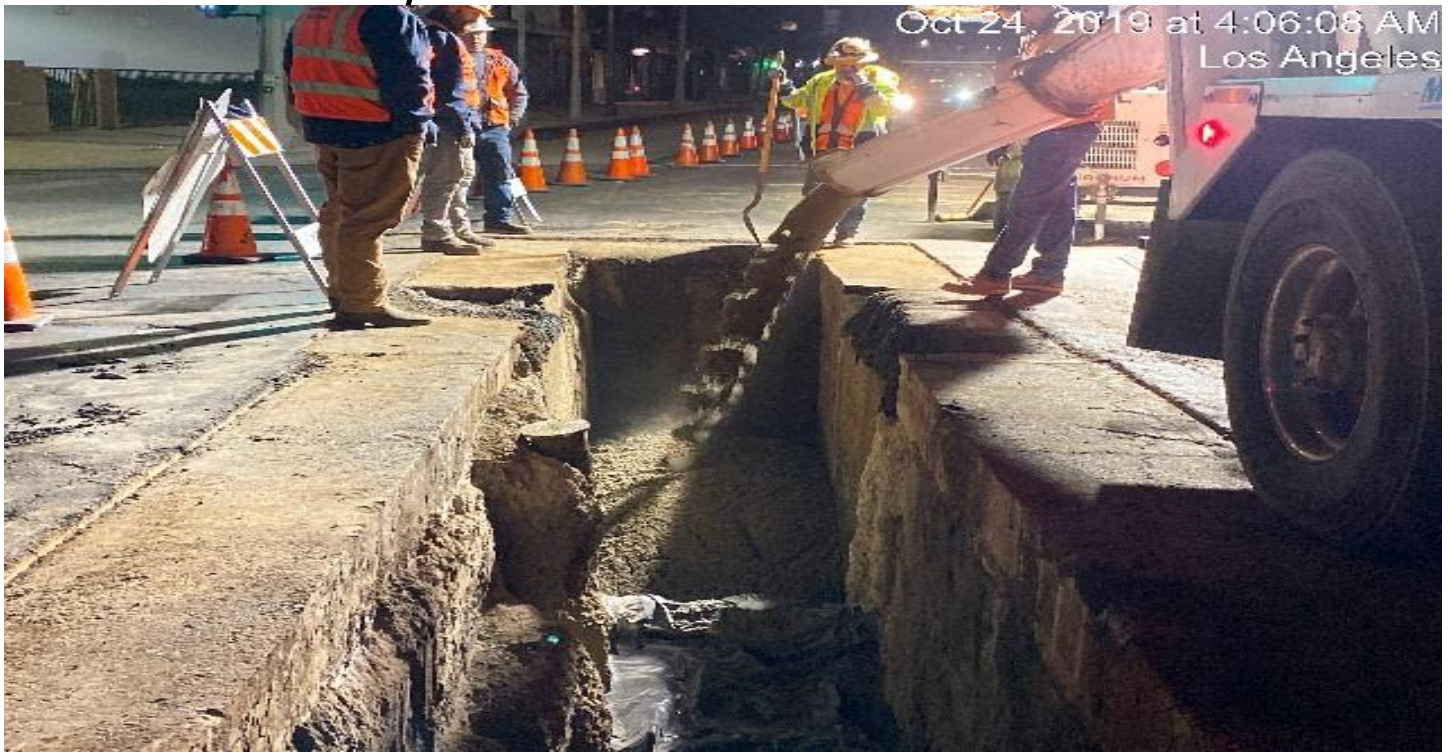
LEIMERT PARK STATION- Placing case 5 encasement for W – Line storm drain on the intersection of 43rd St & Crenshaw Blvd.
