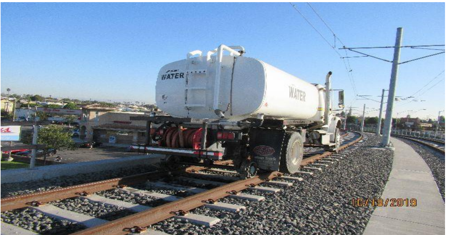
FLORENCE/LA BREA- HCC secured hi-rail water truck on #3 SB track south side of La Brea OP.
