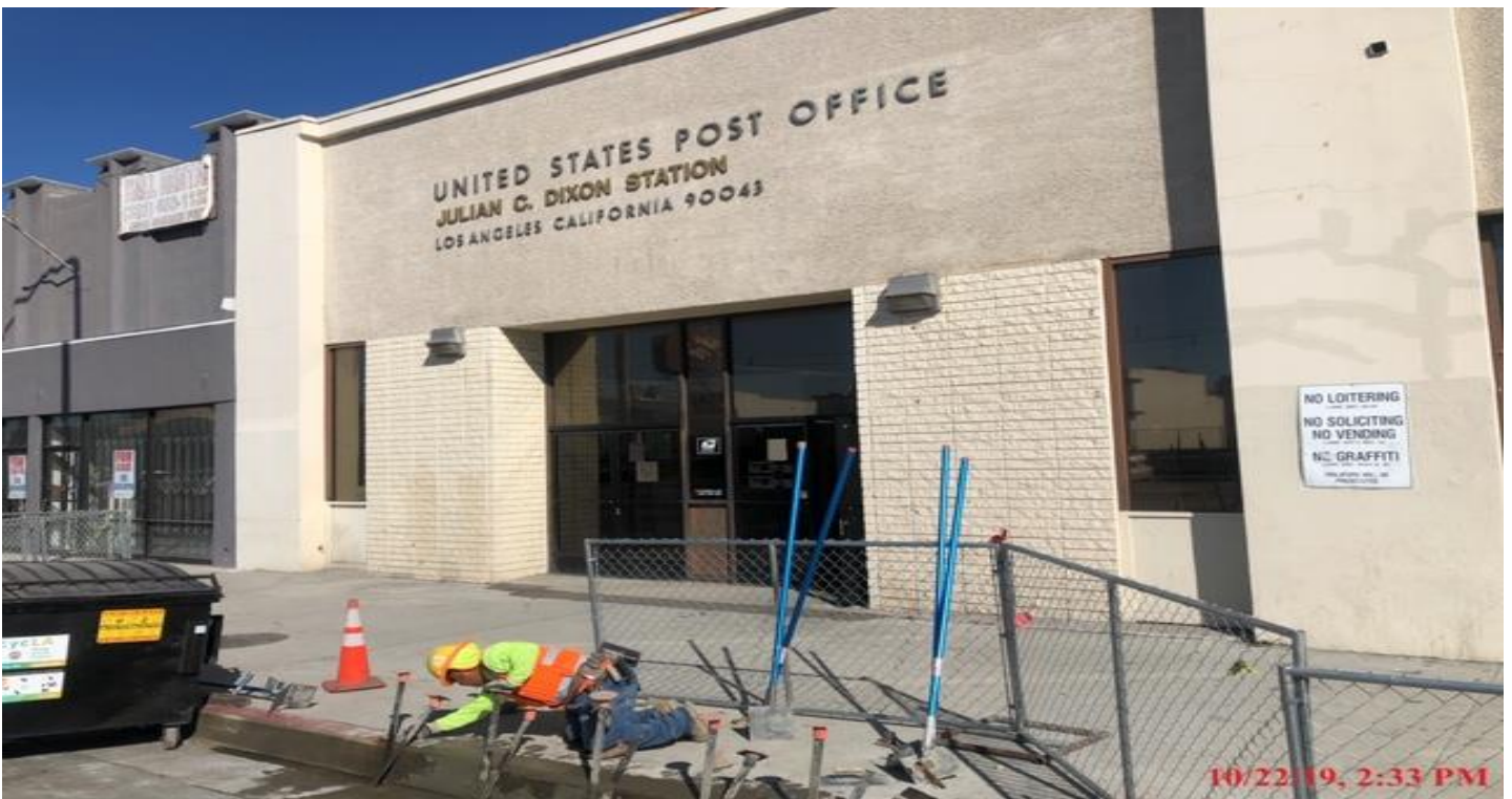
PARK MESA- Curb and gutter placement on the northbound side of Crenshaw Blvd from 54th to 57th St.
