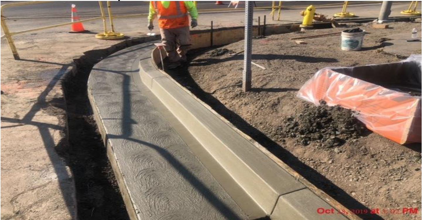
PARK MESA- Curb and gutter placement on the northeast corner of 66th Pl & Crenshaw Blvd.
