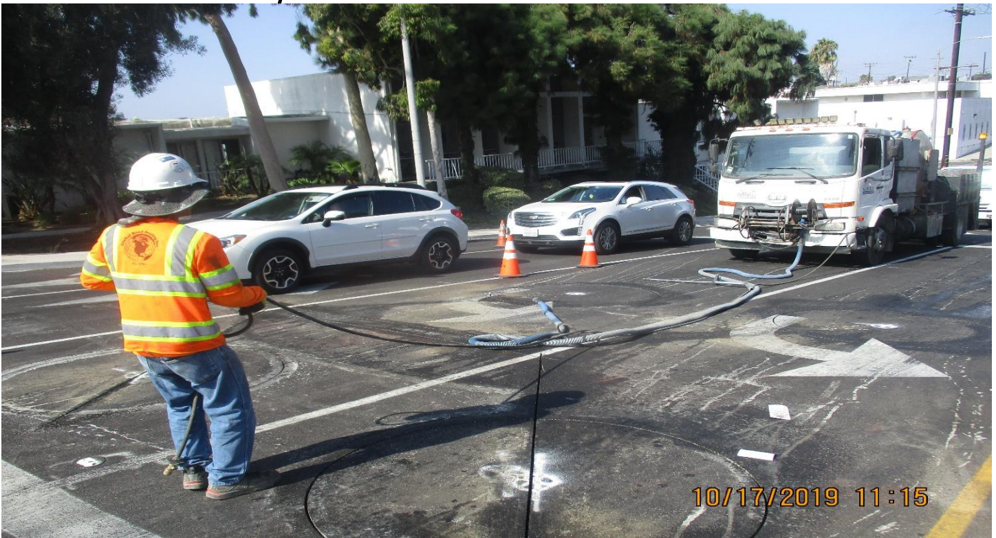
CENTINELA AVE - GRSI Cutting and placing wire in loops on Centinela St intersection.
