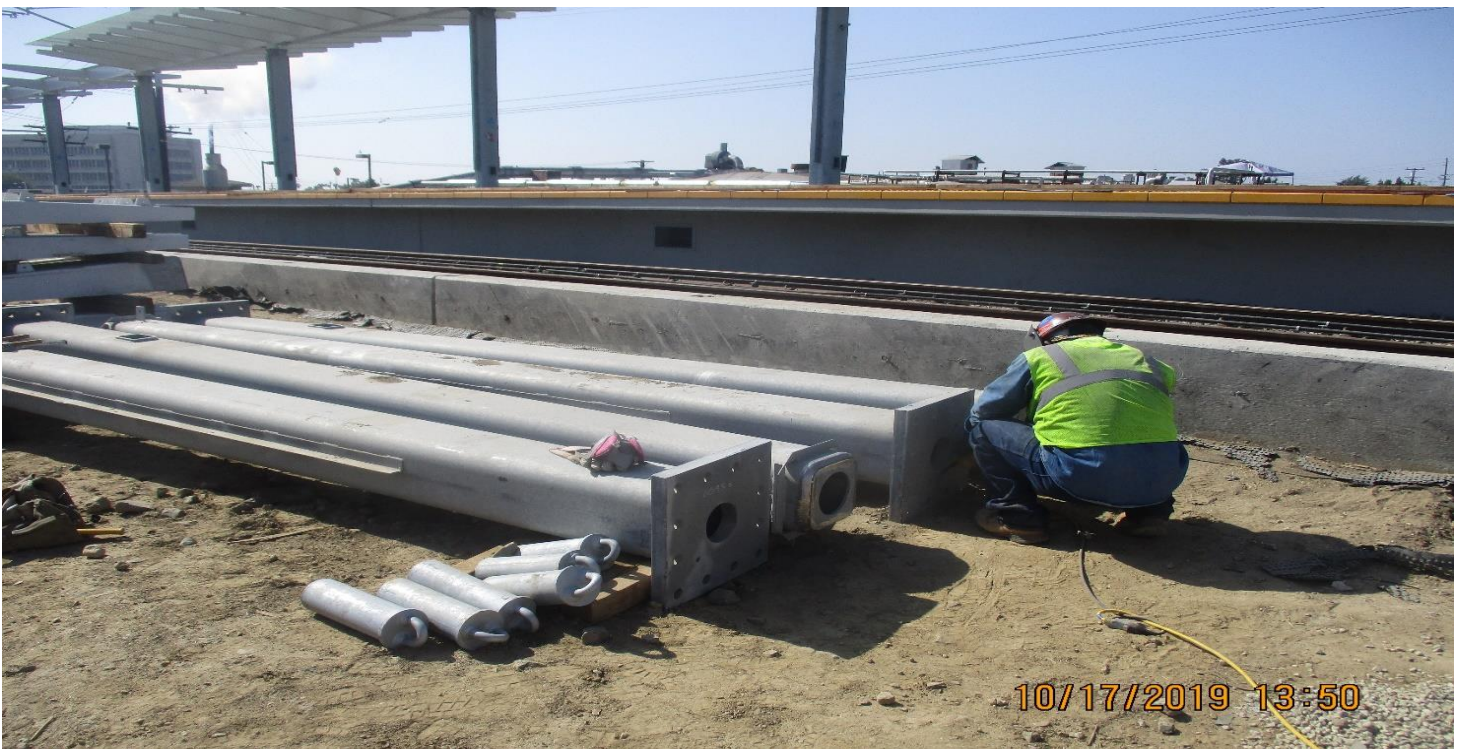
FLORENCE/LA BREA- McMahon Work on ticket plaza columns at La Brea Station.
