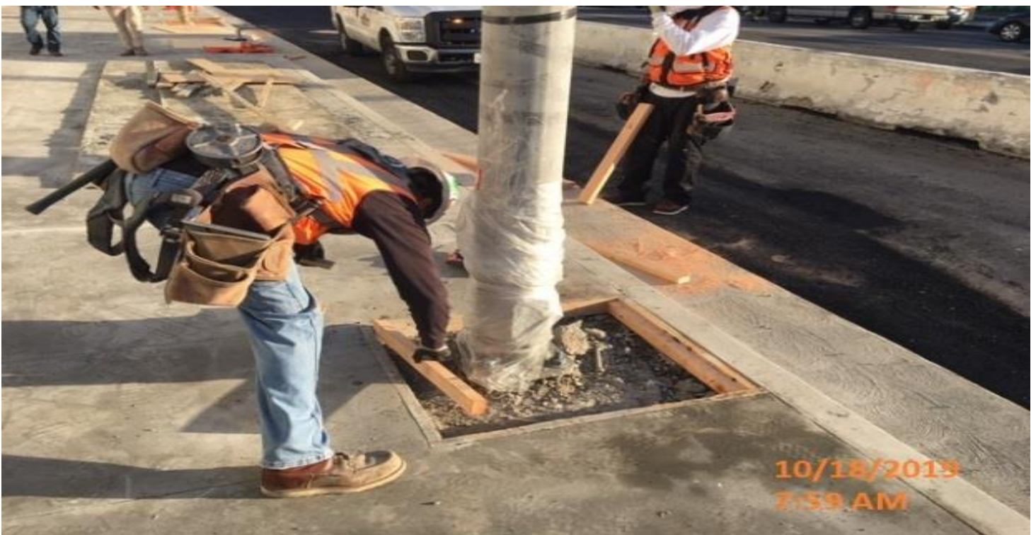
EXPOSITION/CRENSHAW STATION – Forming tree wells for sidewalk posts on the southwest corner of Obama Blvd and Crenshaw Blvd.
