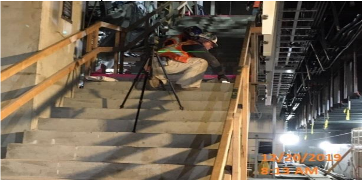
EXPOSITION/CRENSHAW STATION – Laying out installation of granite steps for staircases from concourse to platform level.
