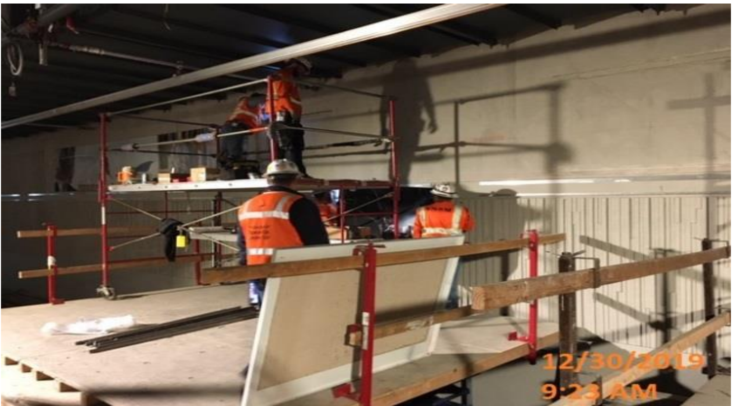
MARTIN LUTHER KING STATION – Continued working on installing the artwork panels along the northbound track of the platform level.
