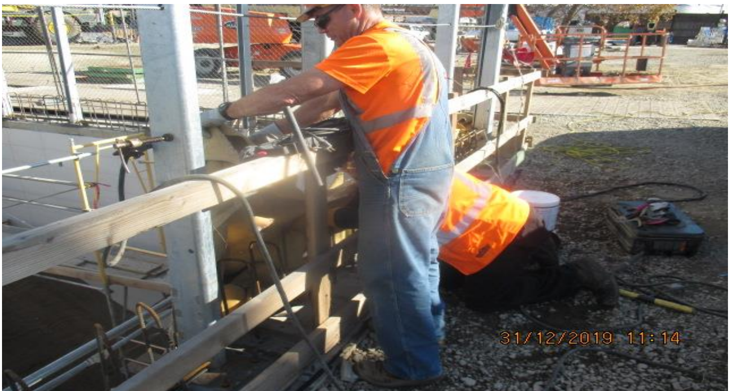
EXPOSITION/CRENSHAW STATION – Continue installing rebar and welding metal wind screen dividers for Elevators 1&2 at the plaza level. 12/31/19
