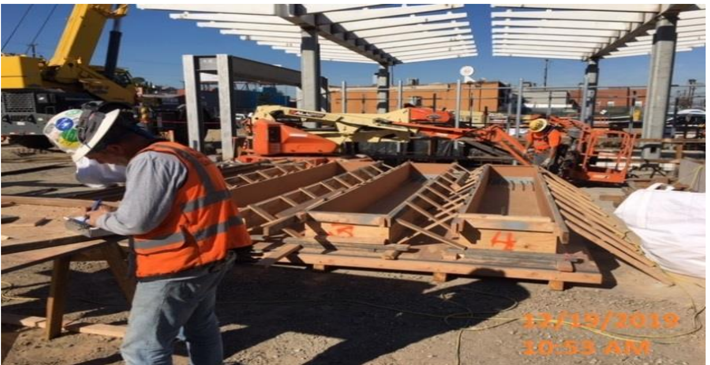
LEIMERT PARK STATION- Continue precast panel formwork for the south equipment access area located at the plaza level.
