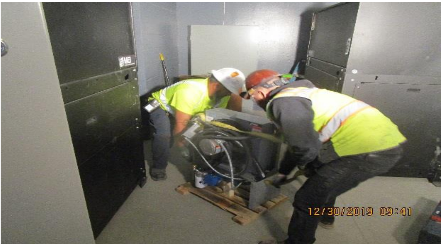
MARTIN LUTHER KING STATION – Setting and anchoring hydraulic power units and controllers in Elevator Machine Room C – 116 at the concourse level.
