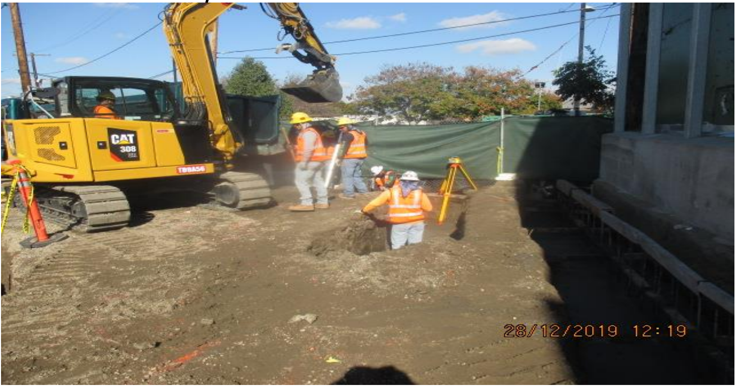
LEIMERT PARK STATION- Continued formwork for plantar wall at the plaza level. 12/28/19
