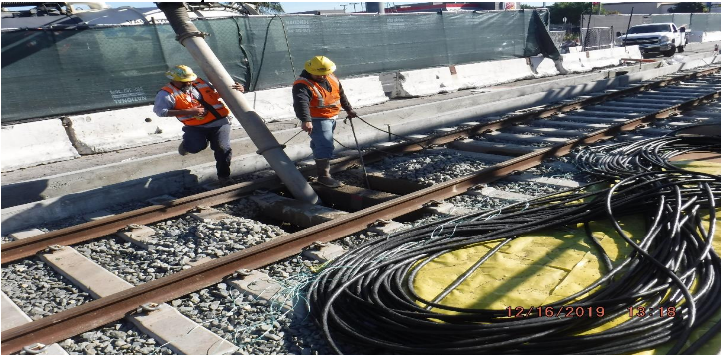
B2 GUIDEWAY - Track ballast disturbance searching for systems conduits near Slauson Station.
