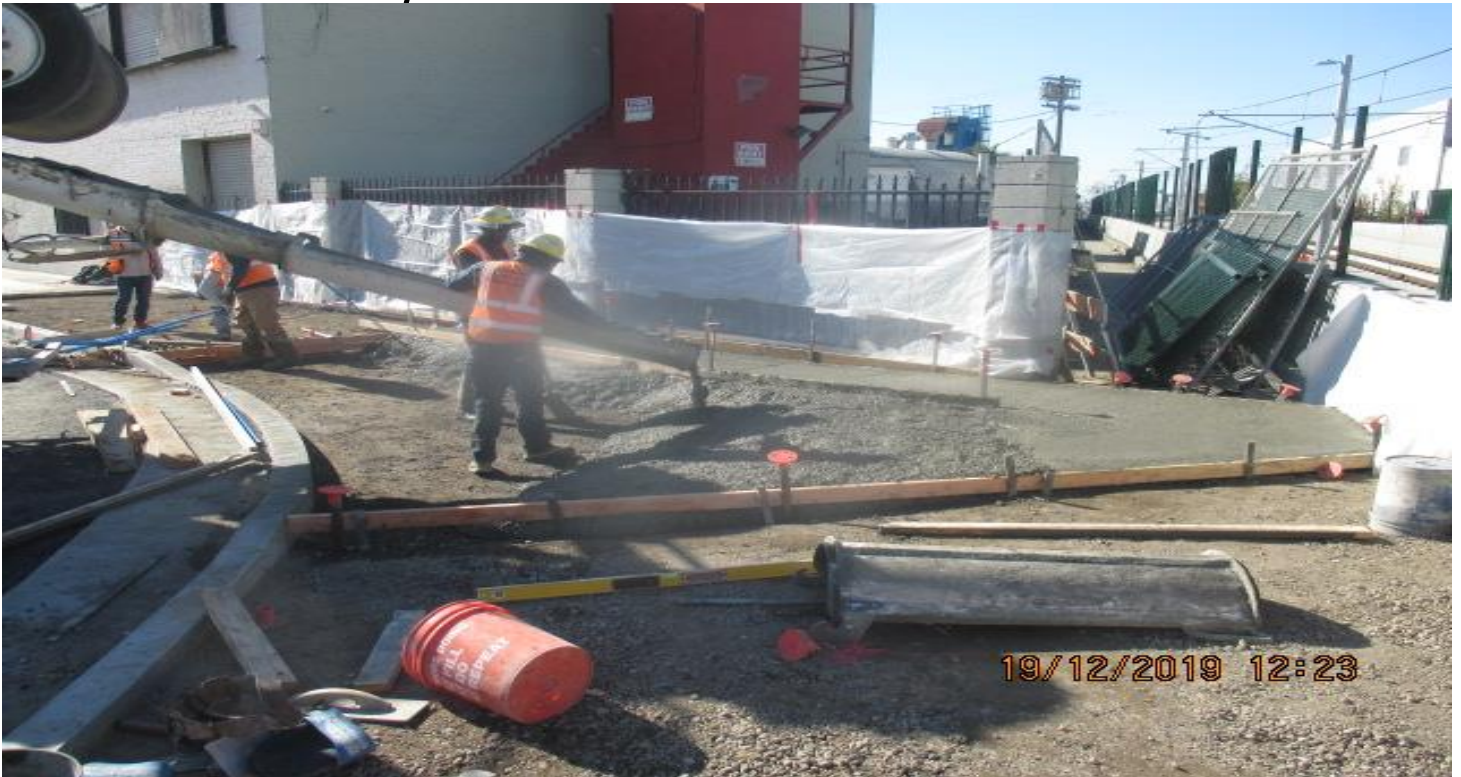
UG3- Forming and placing concrete for the pedestrian ramp on the southbound side of Victoria Ave. 12/19/19
