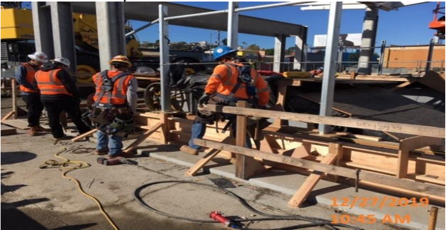
LEIMERT PARK STATION- Continued formwork for the wind screen curbs on the main entrance canopy at the plaza level.
