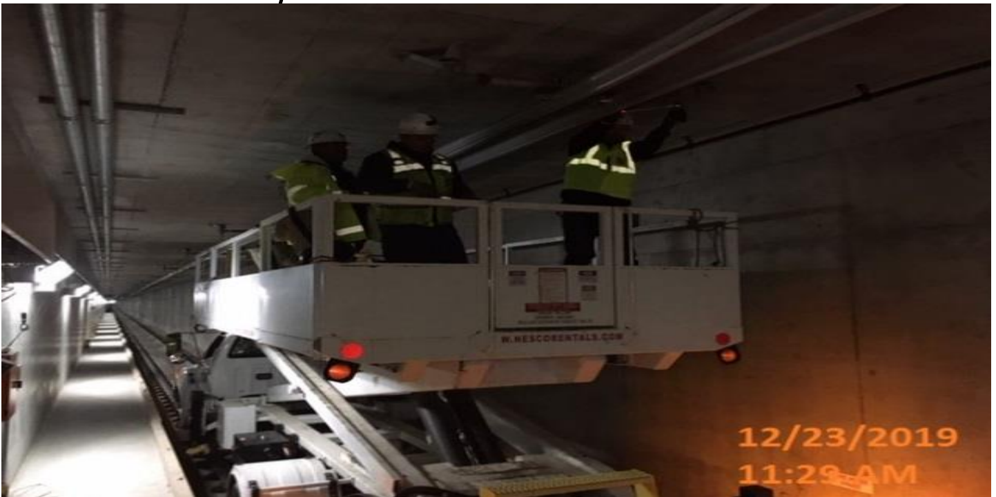
UG3- Registering and staggering the overhead contact system along the northbound tunnel at Sta 287+85.
