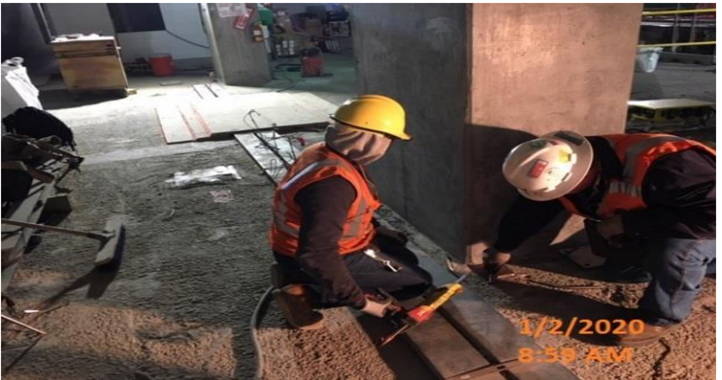
MARTIN LUTHER KING STATION – Setting base plates for the fare collection system at the concourse level.
