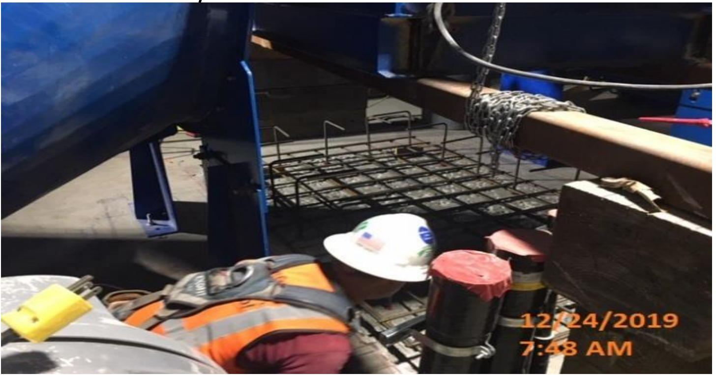
EXPOSITION/CRENSHAW STATION – Adjusting rebar form the emergency ventilation fan pads in the South Fan Rooms of the concourse level.
