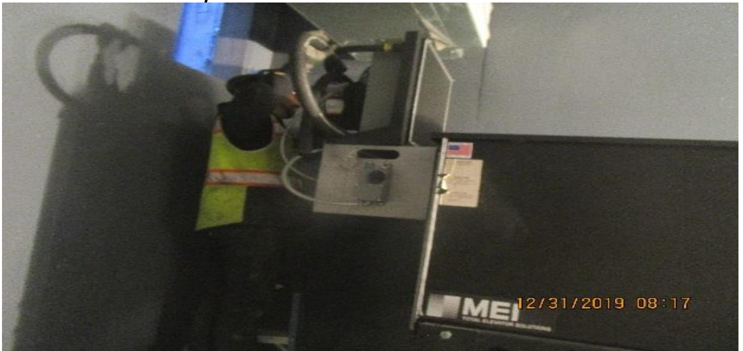
MARTIN LUTHER KING STATION – Continue setting and anchoring hydraulic power units and oil coolers in Elevator Machine Room C – 116 at the concourse level.
