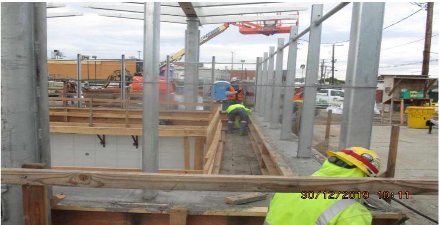
LEIMERT PARK STATION- Stripping formwork for the wind screen curbs on the main entrance canopy at the plaza level. 12/30/19.
