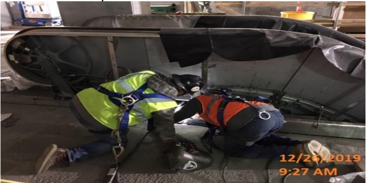
MARTIN LUTHER KING STATION – Installing bent plates at the edge slab of Escalator #4 at the concourse level.
