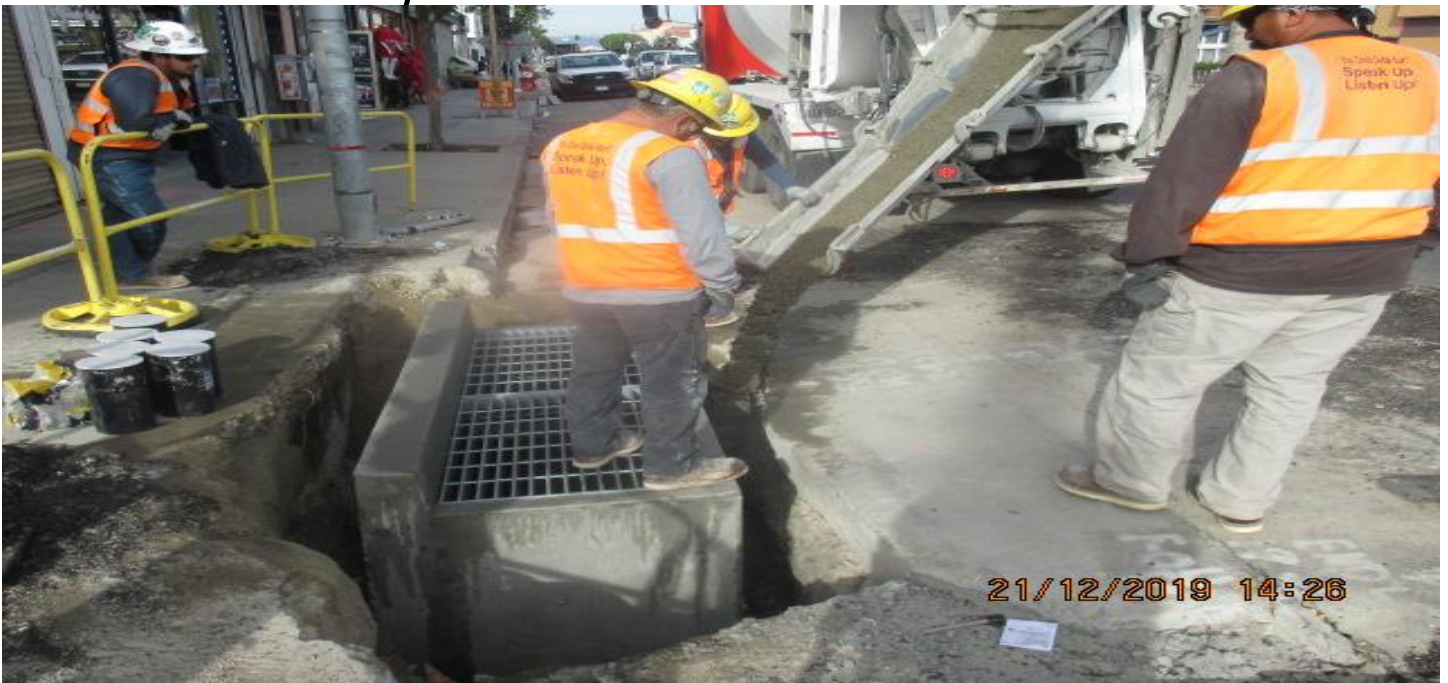
PARK MESA- Placing concrete for Catch Basin #2 located on the northwest corner of Hyde Park Blvd & Crenshaw Blvd. 12/21/19.
