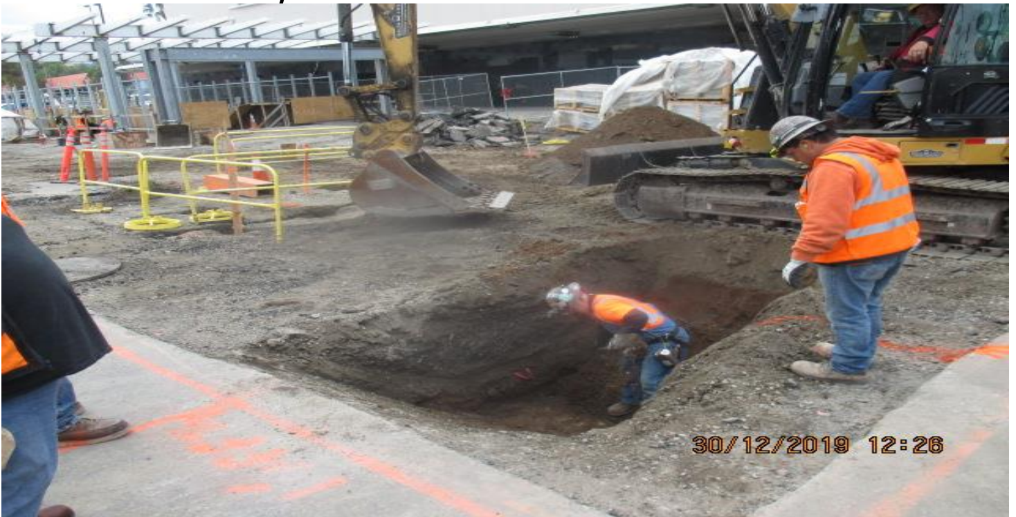
MARTIN LUTHER KING STATION – Excavation for reinforced concrete pipe placement for W – Line storm drain on the northwest corner of Obama Blvd and Crenshaw Blvd.
