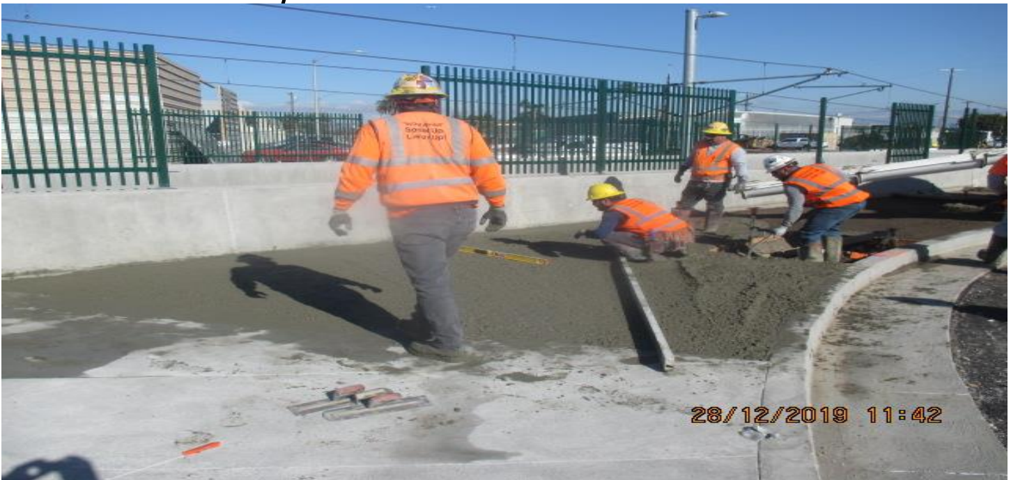
UG3- Continued placing concrete for the pedestrian ramp on the southbound side of Victoria Ave. 12/28/19
