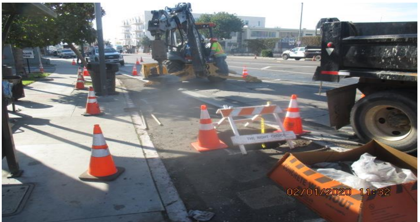
PARK MESA – Excavation of sidewalk for street and signal lights on the southeast corner of 60th St & Crenshaw Blvd. 2/1/20
