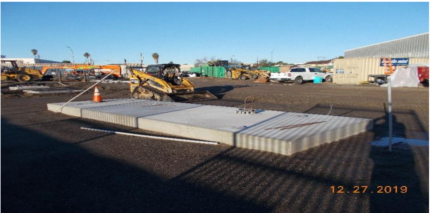
UG3- Backfilling and compacting soil for the auxiliary power site at Victoria Yard adjacent to the south end portal. (No change since last update)
