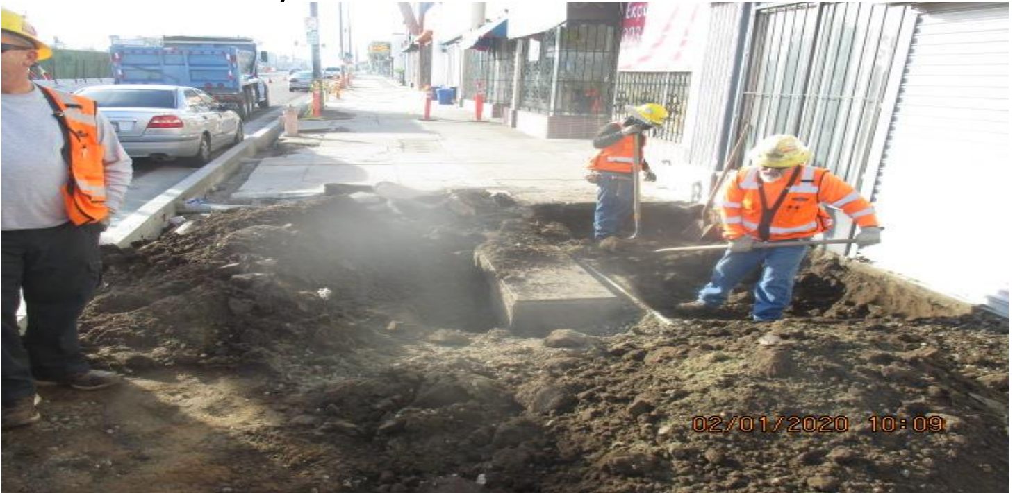
PARK MESA – Continued sidewalk excavation on Crenshaw Blvd from Brynhurst Ave to 48th St. 1/2/20
