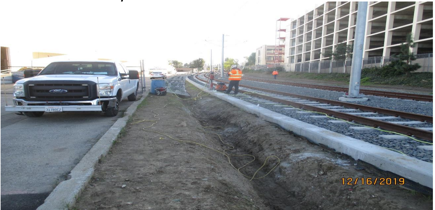
B1 GUIDEWAY – Coring fence post holes in ballast wall near FCBC at Eucalyptus.
