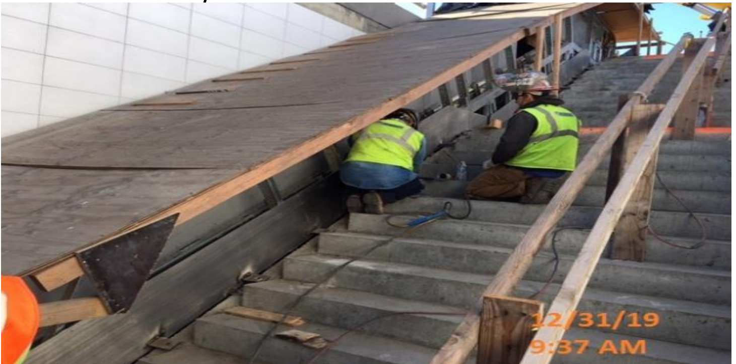
LEIMERT PARK STATION - Continue welding edge plates to Escalator 1&2 at the main staircase landing between the plaza and intermediate levels.
