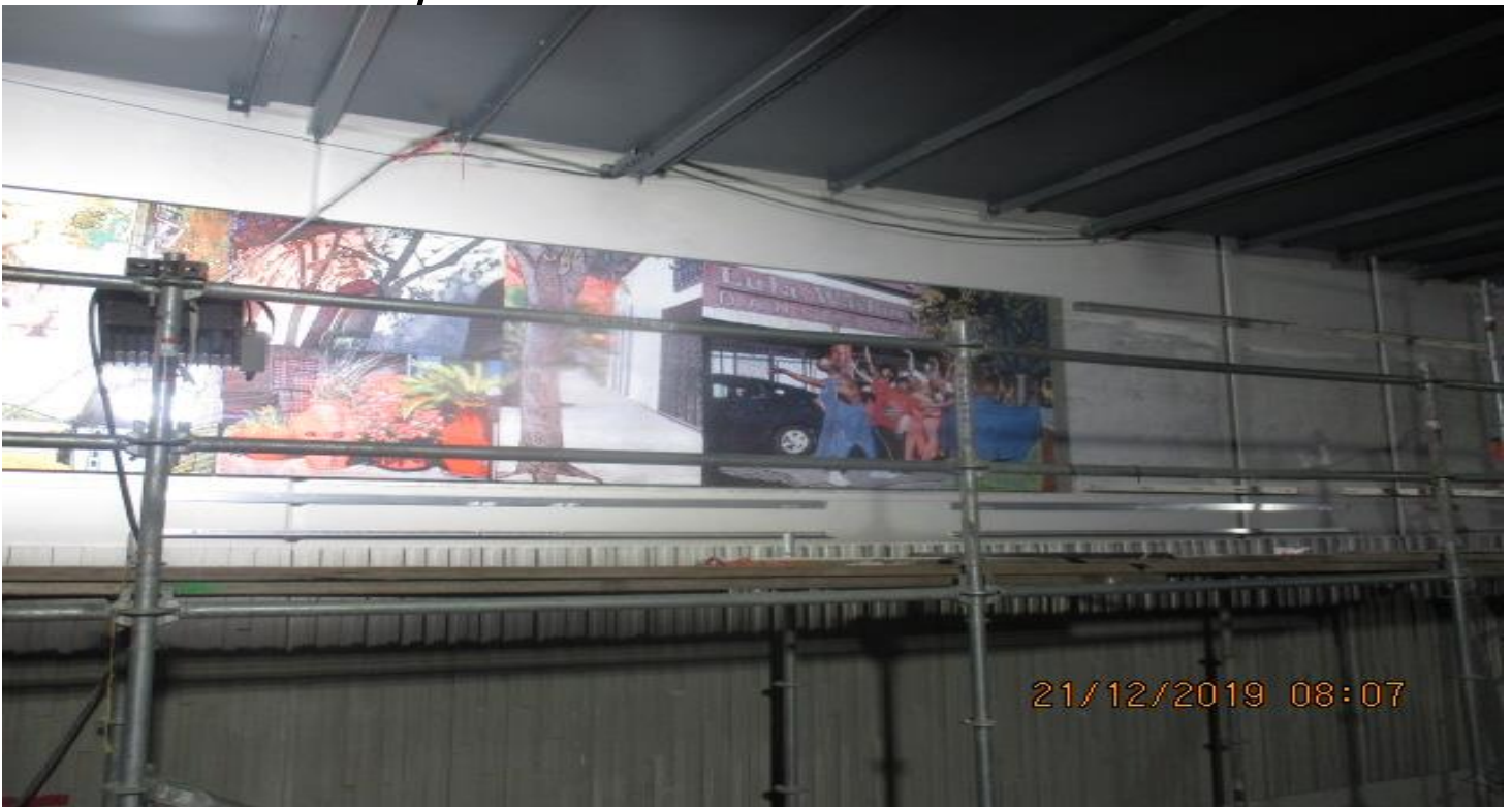
EXPOSITION/CRENSHAW STATION – Installation of angle brackets and porcelain enamel art panels on the northbound track of the platform level. 12/21/19
