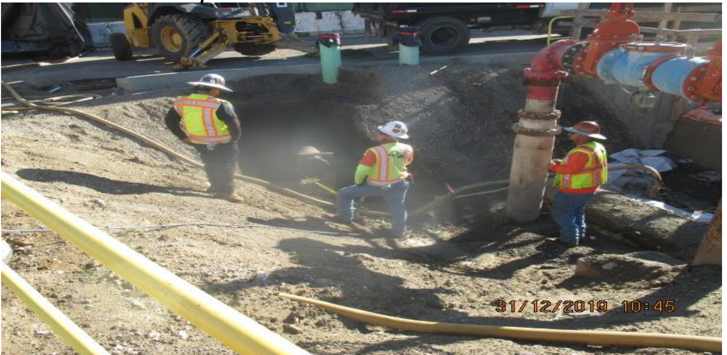
MARTIN LUTHER KING STATION – Excavating for the extension of the 8” fire department connection at the plaza level. 12/31/19.
