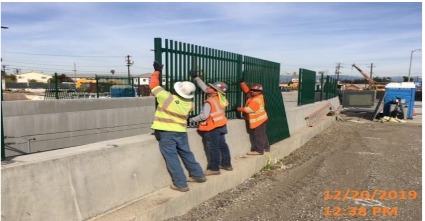
UG3- Continued installation of fence posts and panels on the north and southbound track walls from Sta 279+47 to 282+00.
