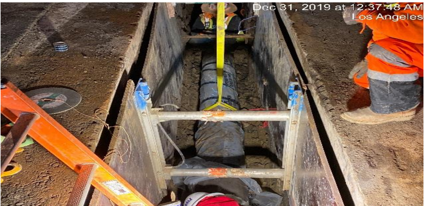
PARK MESA- Laying pipe and slurry for 12" LADWP service line on the intersection of 60th St & Crenshaw Blvd.
