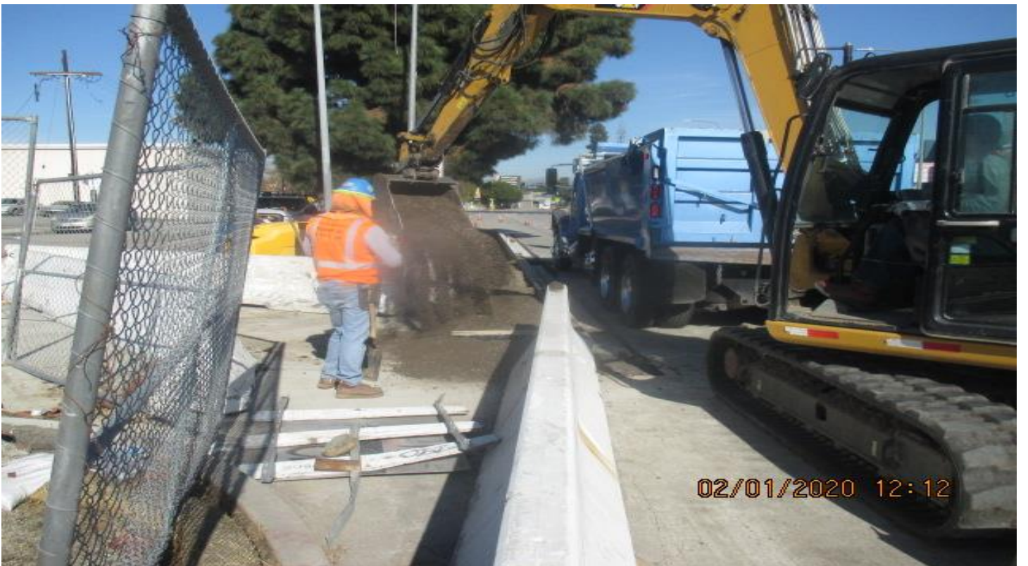
LEIMERT PARK STATION- Placing backfill and compacting sidewalk on northbound Leimert Blvd and Crenshaw Blvd. 1/2/20
