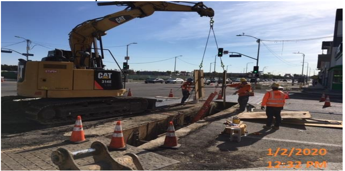
EXPOSITION/CRENSHAW STATION – Laying 24” of concrete reinforced pipe for Line U – storm drain on the northwest corner of Rodeo Blvd and Crenshaw Blvd.
