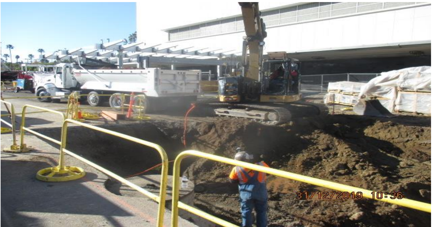
MARTIN LUTHER KING STATION – Continue excavating for the installation of the oil water separator at the plaza level. 12/31/19.
