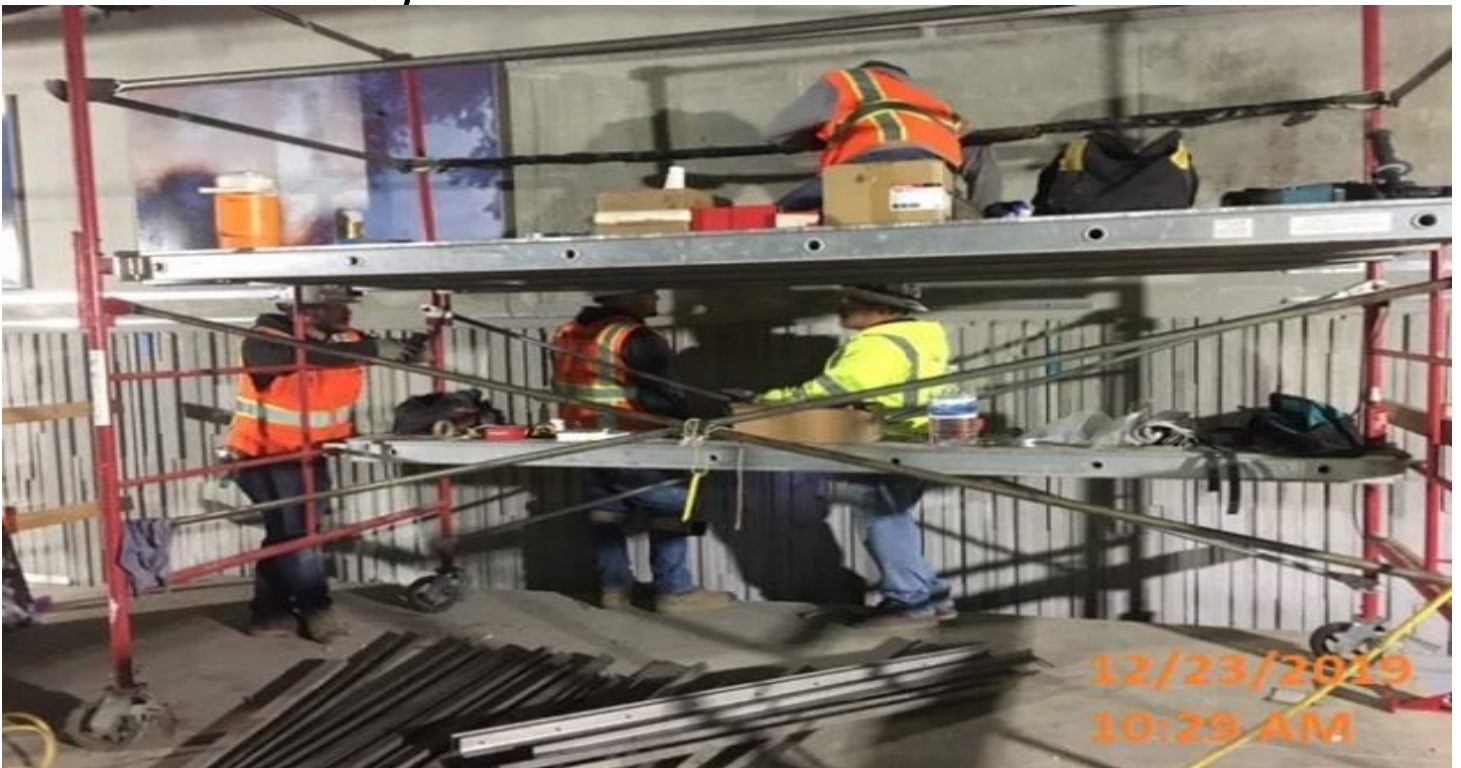
LEIMERT PARK STATION - Continued installation of porcelain enamel art panel on the northbound track of the platform level.
