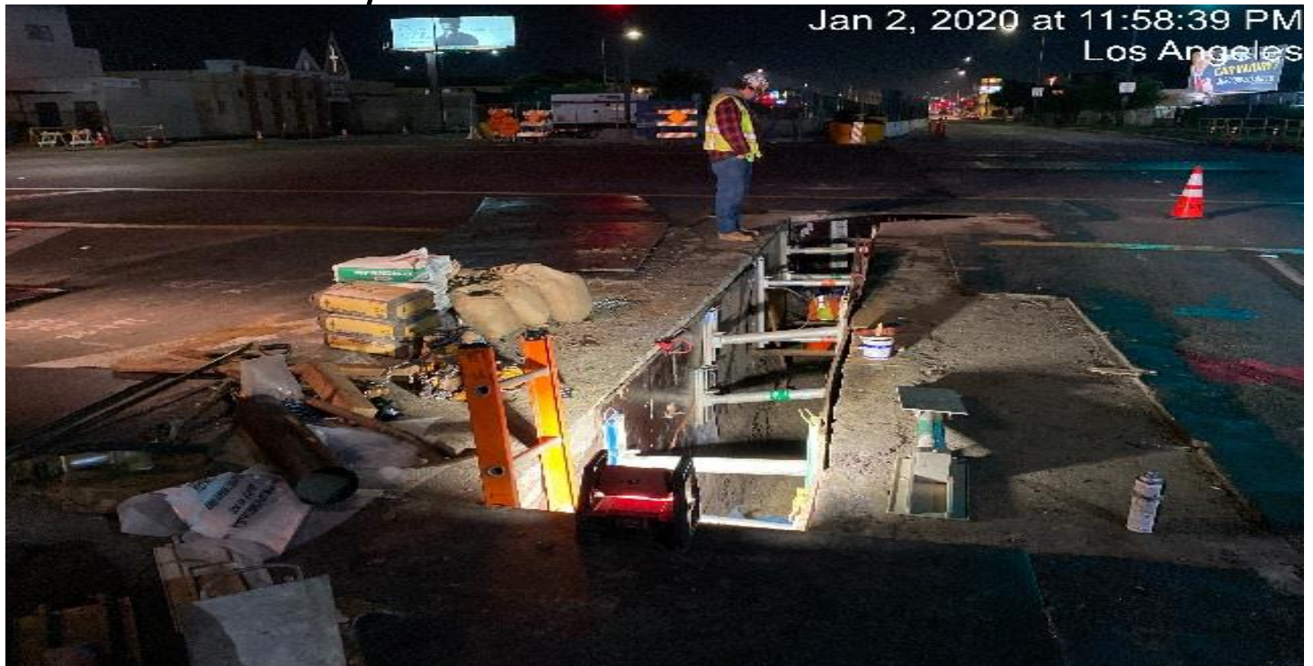
PARK MESA – Continue laying pipe and slurry for 12” LADWP service line on the intersection of 60th St & Crenshaw Blvd.
