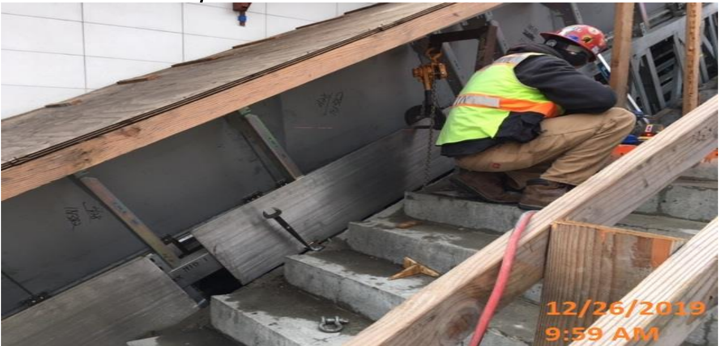
LEIMERT PARK STATION - Installing edge plates to Escalator 1&2 at the main staircase landing between the plaza and intermediate levels.
