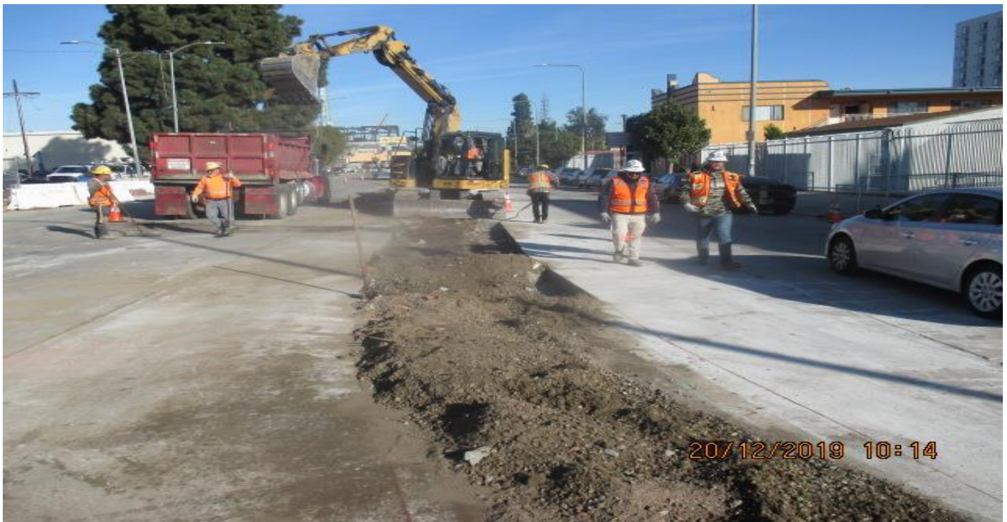
LEIMERT PARK STATION- Continue saw cutting and excavating both sides of center median divider at northbound Leimert Blvd and Crenshaw Blvd. 12/20/19
