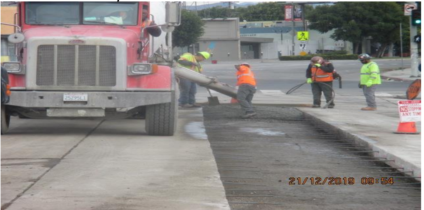
LEIMERT PARK STATION- Continue excavating and placing concrete on the center median divider at northbound Leimert Blvd and Crenshaw Blvd. 12/21/19
