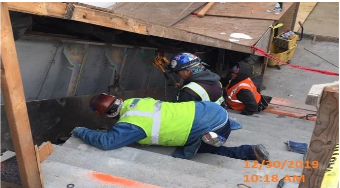
LEIMERT PARK STATION - Continue installing edge plates to Escalator 1&2 at the main staircase landing between the plaza and intermediate levels.
