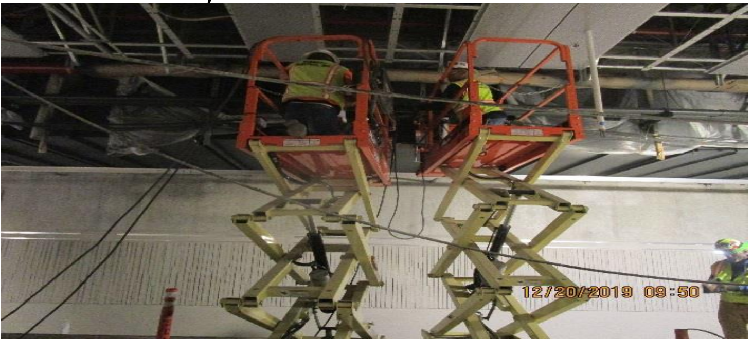
MARTIN LUTHER KING STATION – Continued setting and welding edge lighting support posts #5 of 18 imbeds at the southbound track of the platform level.
