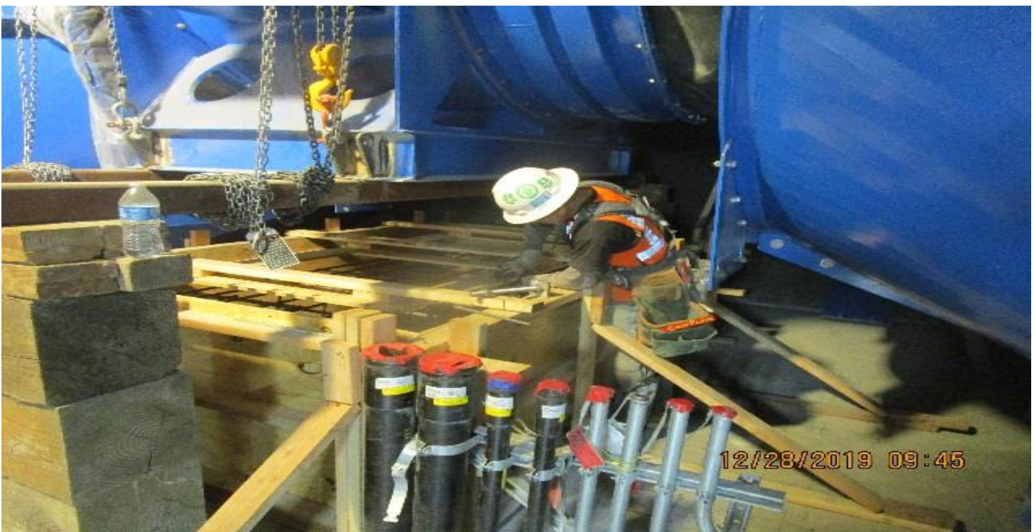
EXPOSITION/CRENSHAW STATION – Installing anchor bolts to emergency ventilation fan foundation pad in the North Fan Room of the concourse level.
