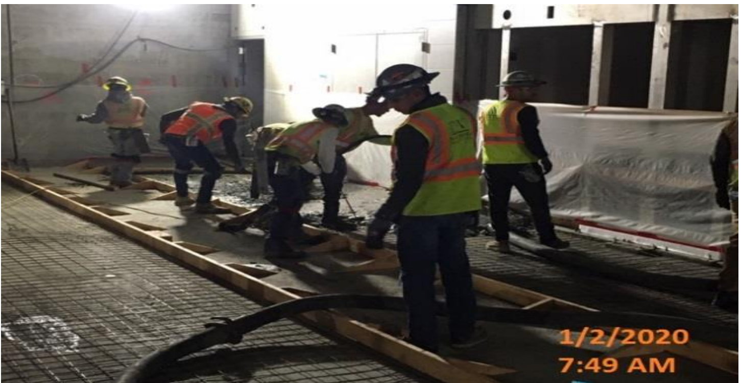
EXPOSITION/CRENSHAW STATION – Placing remaining concrete for the architectural topping slab at the concourse level.
