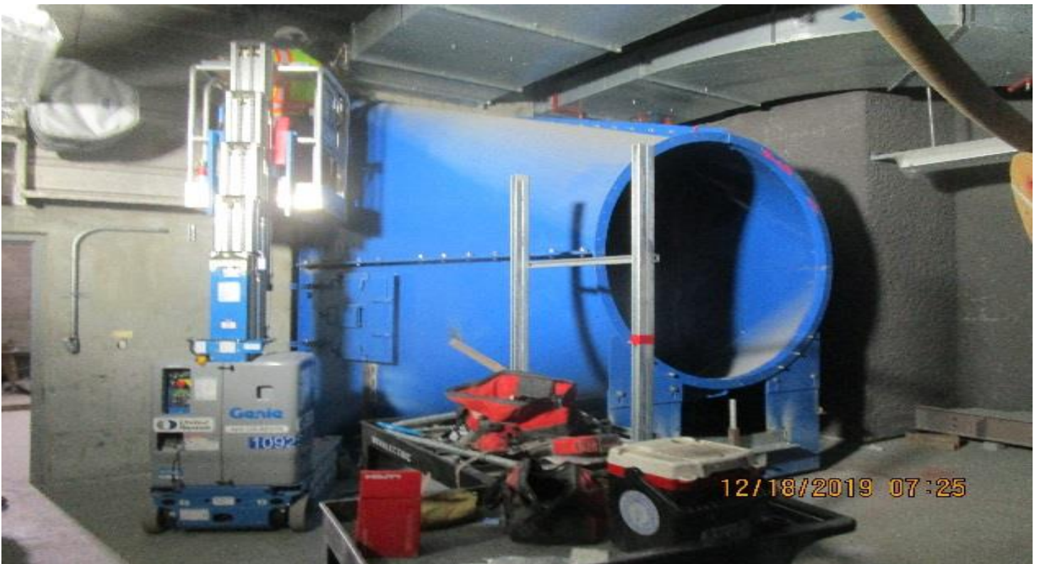
LEIMERT PARK STATION - Rerouting fit up for square to round transition pieces of the emergency ventilation fan units in the North Fan Room of the concourse level.
