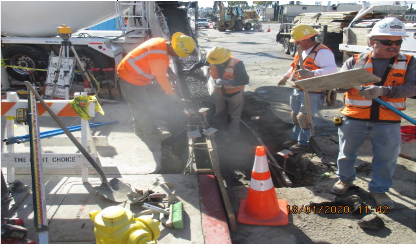
UG3 – Continued new curb/gutter and ADA ramp installation on the northeast corner of 67th St and Crenshaw Blvd. 1/18/20
