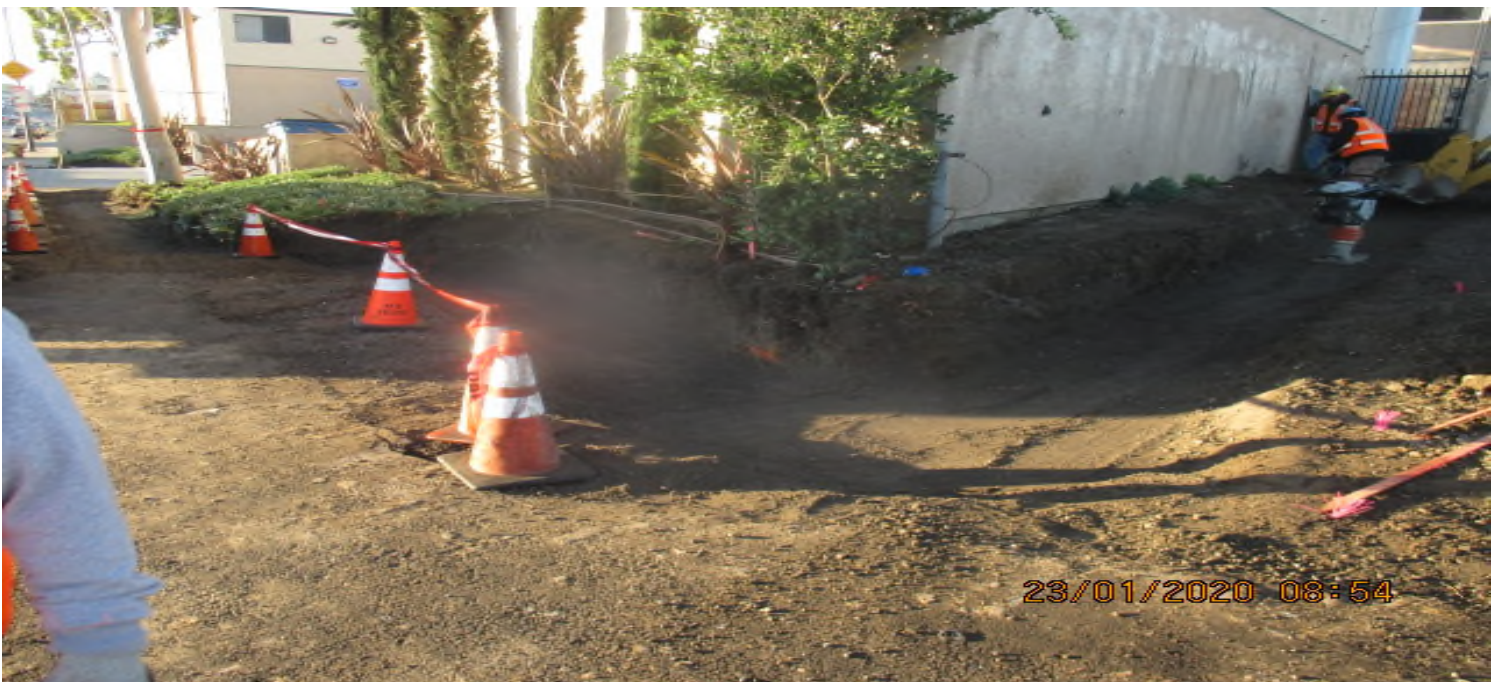
UG3 – Excavation for the southwest sidewalk curb of “New Road” at the intersection of Crenshaw Blvd. 1/23/20.
