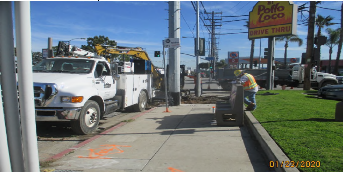
Aviation/Century – Sidewalk demo on the south east corner of Manchester and Aviation.
