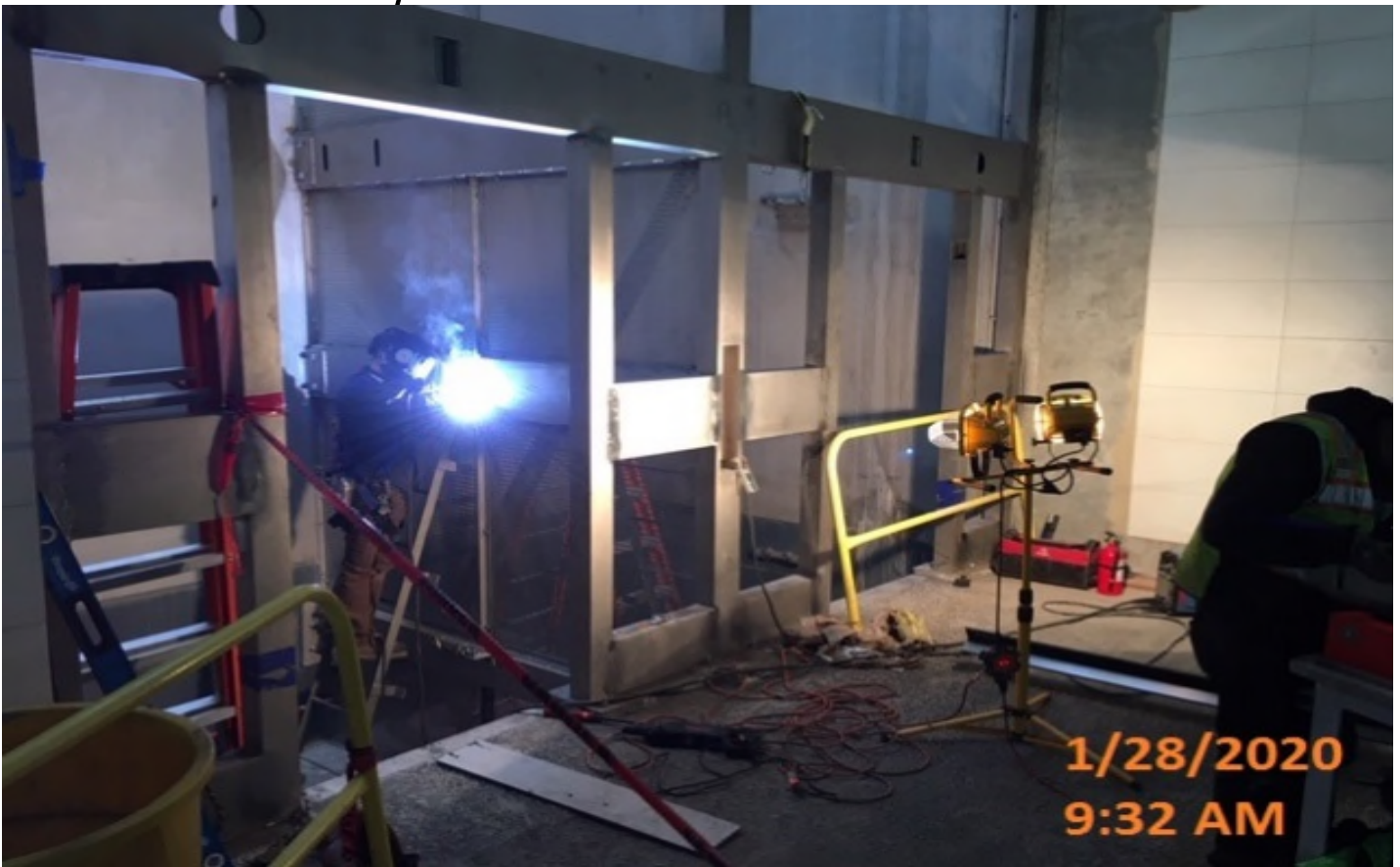
MLK Station - Continued jack installation and began welding starter rail brackets inside Elevator shafts 1&2 at the concourse level.
