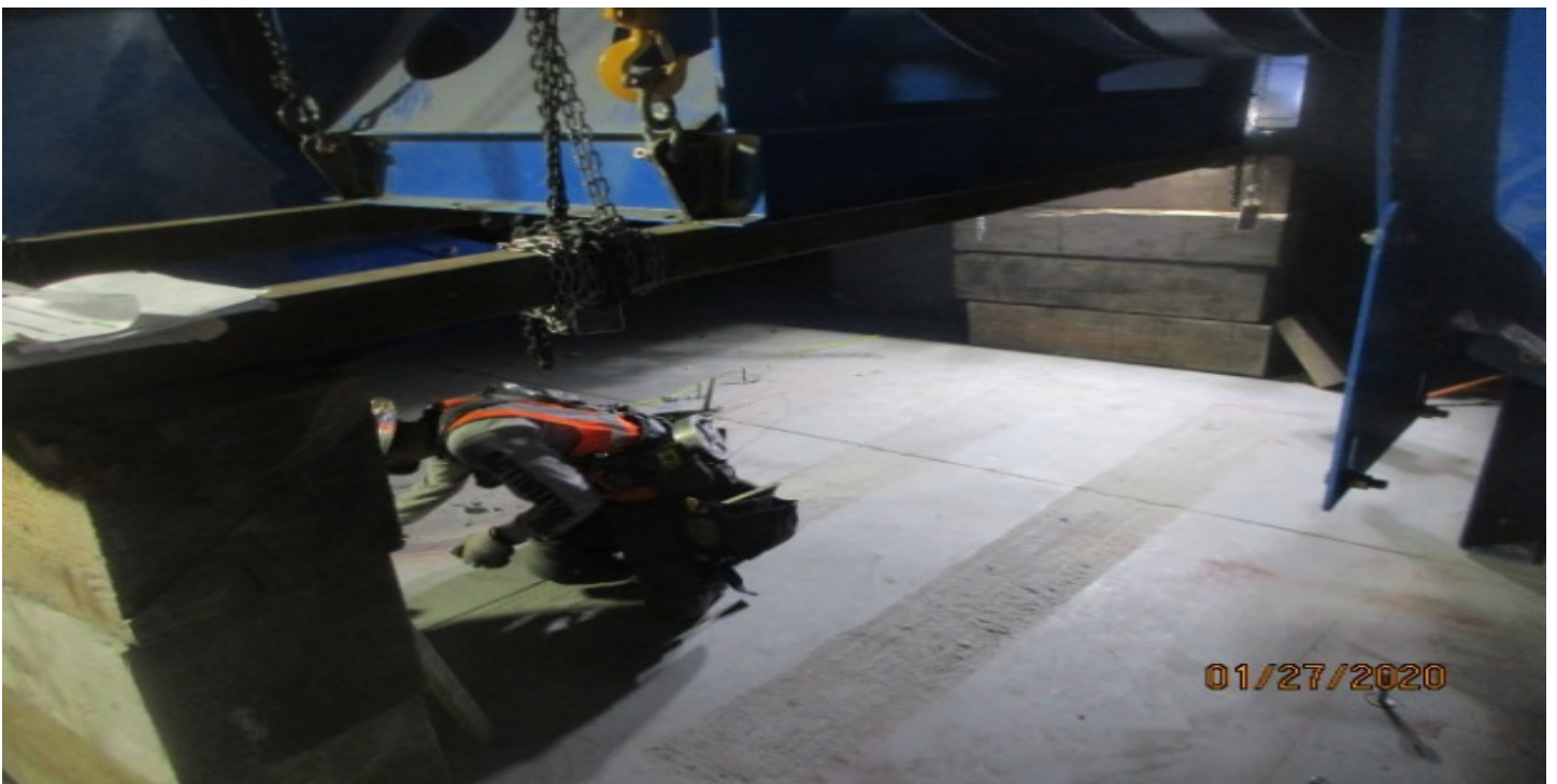
MLK Station - Scanning and drilling dowels for EVF-7-122 and EVF-322 equipment pads in the North Fan Room C – 142 of the concourse level.
