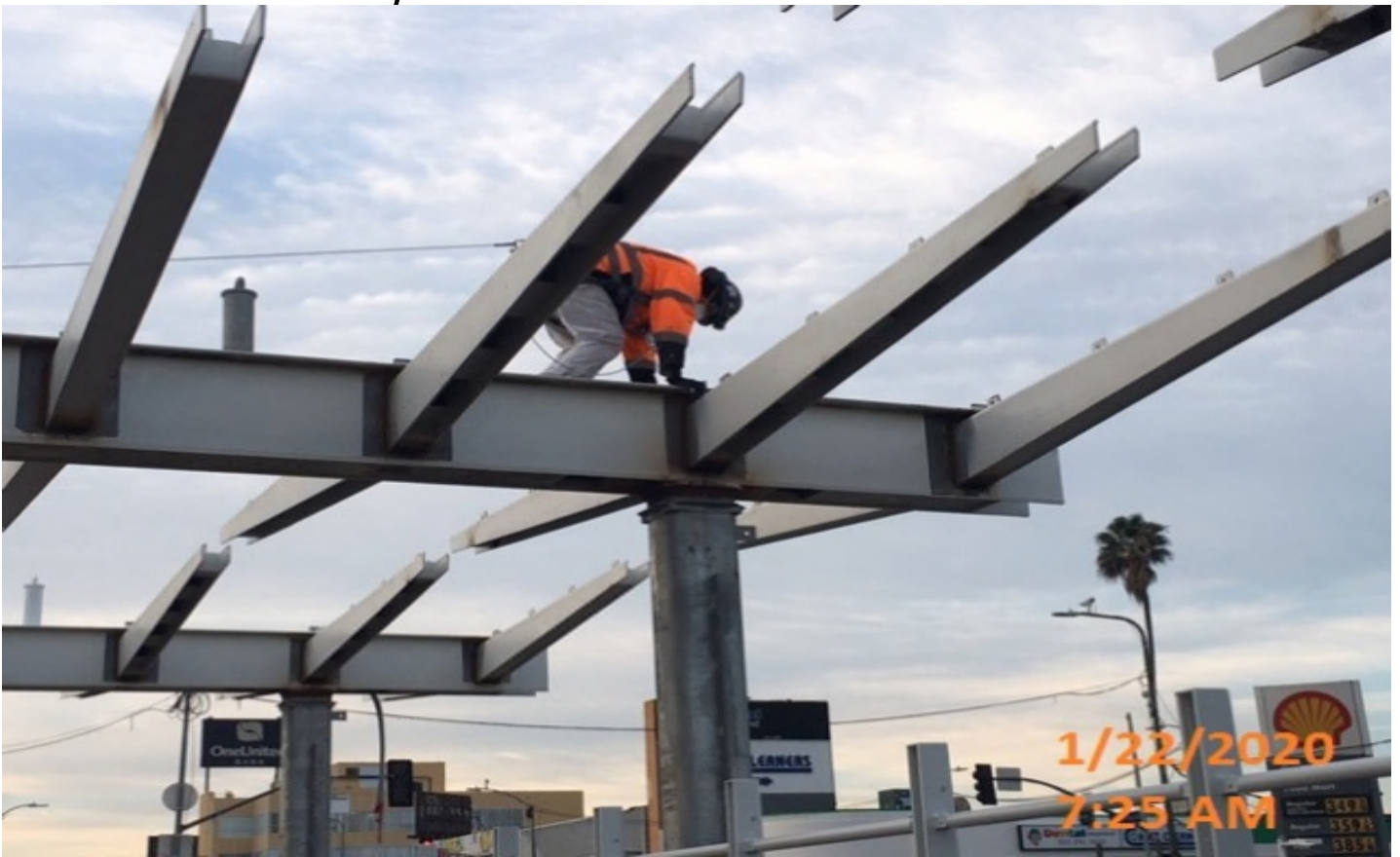
Expo Station - Applying second coat of paint to the wind screen curbs and preparing to prime the main entrance canopy at the plaza level.
