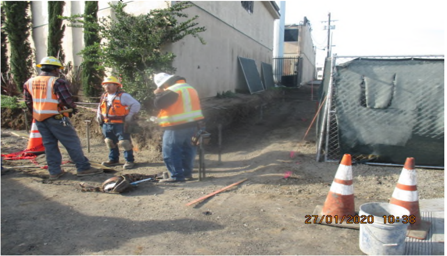
UG3 – Building curb/gutter forms for southwest corner of “New Road” at the intersection of Crenshaw Blvd. 1/27/20
