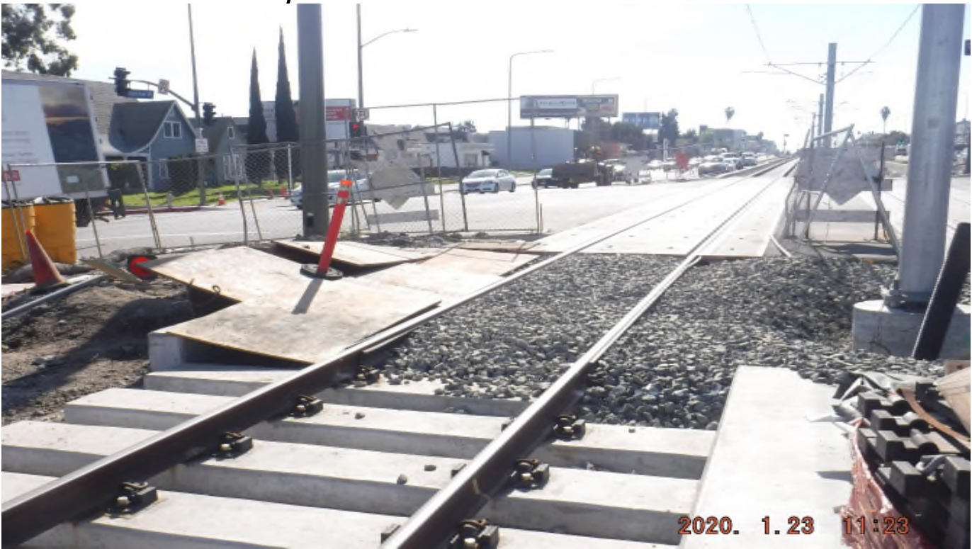
48 th Street - STA364+46_ Looking South_ Track structure disturbance in search of BLS conduits_ 48ST.
