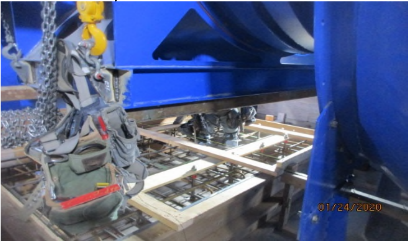
MLK Station - Prepping for concrete placement of EVF-7-121 and 7-321 equipment pads in the South Fan Room C – 102 of the concourse level.
