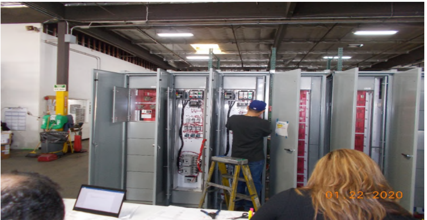
UG - 1 – RESA testing facility - FAT for UG1-MCC
