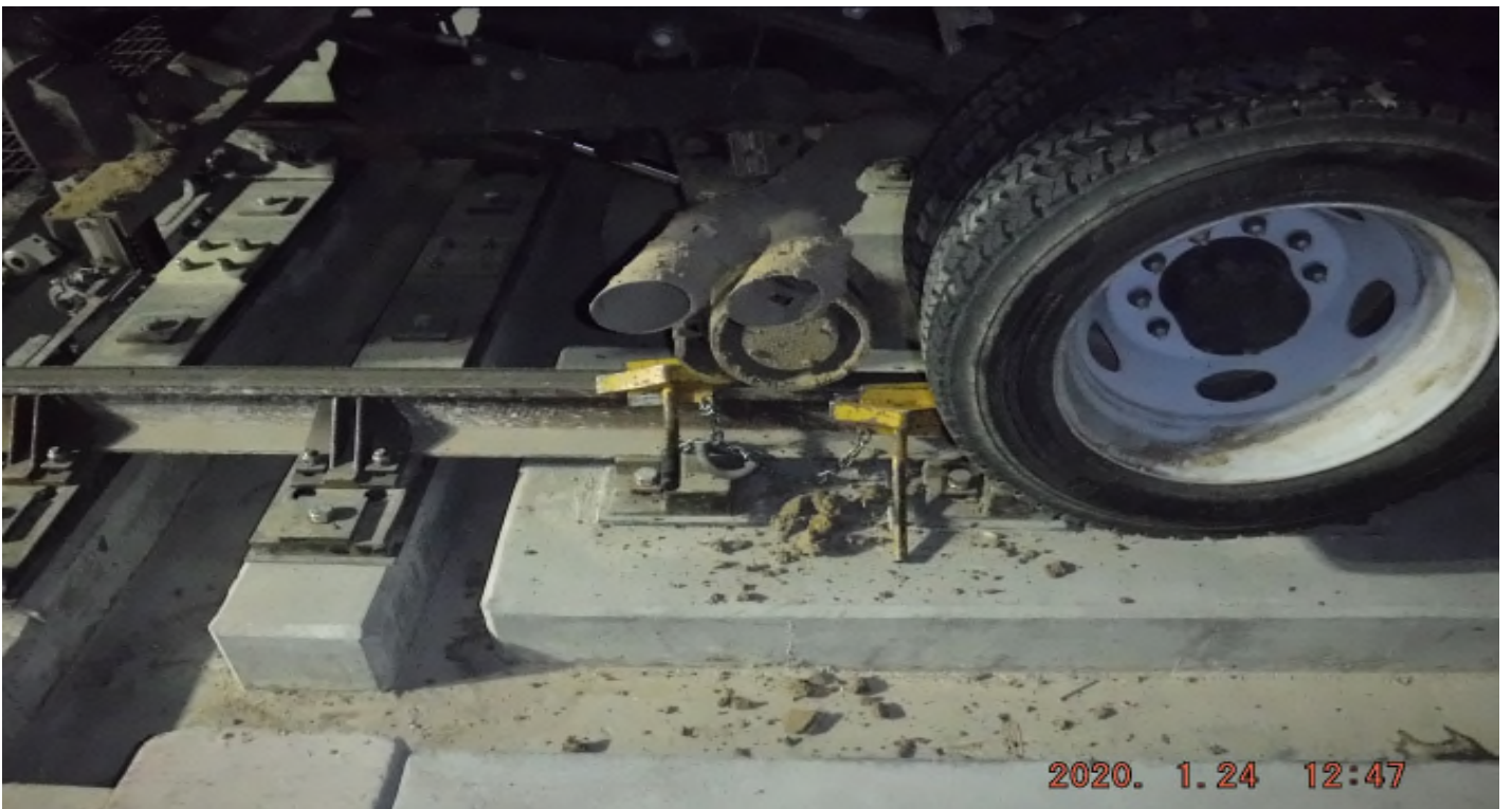
UG-4- STA444+40_ UG4 hi-rail_ Equipment with dirt on Expo invert
