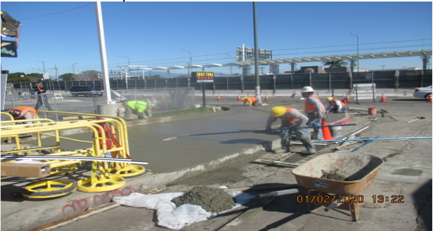
Hyde Park Station – Placing concrete for new curb/gutter, sidewalk and ADA ramp on the north and southwest corners of 58th St & Crenshaw Blvd. 2/1/20
