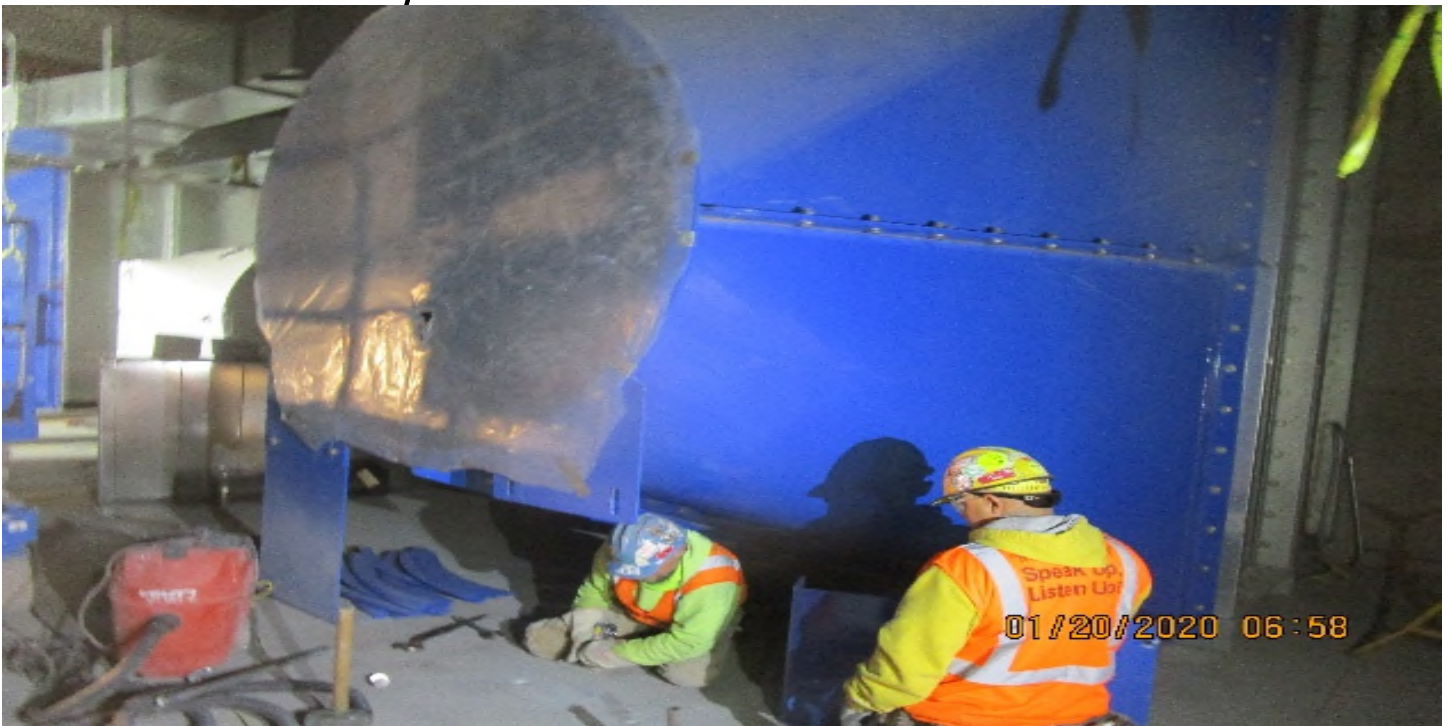
MLK Station - Continue drilling and anchoring EVF-7-122 square to round transition piece in the North Fan Room C – 142 of the concourse level.
