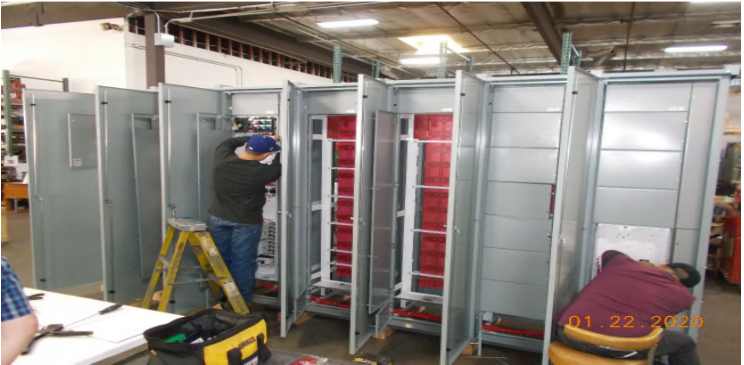
UG - 1 – RESA testing facility - Wiring controls for testing UG1-MCC
