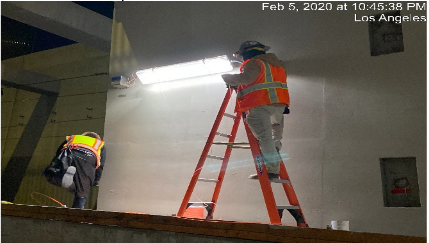
UG3 – Continue pulling wire for the emergency lighting at the south end portal entrance.
