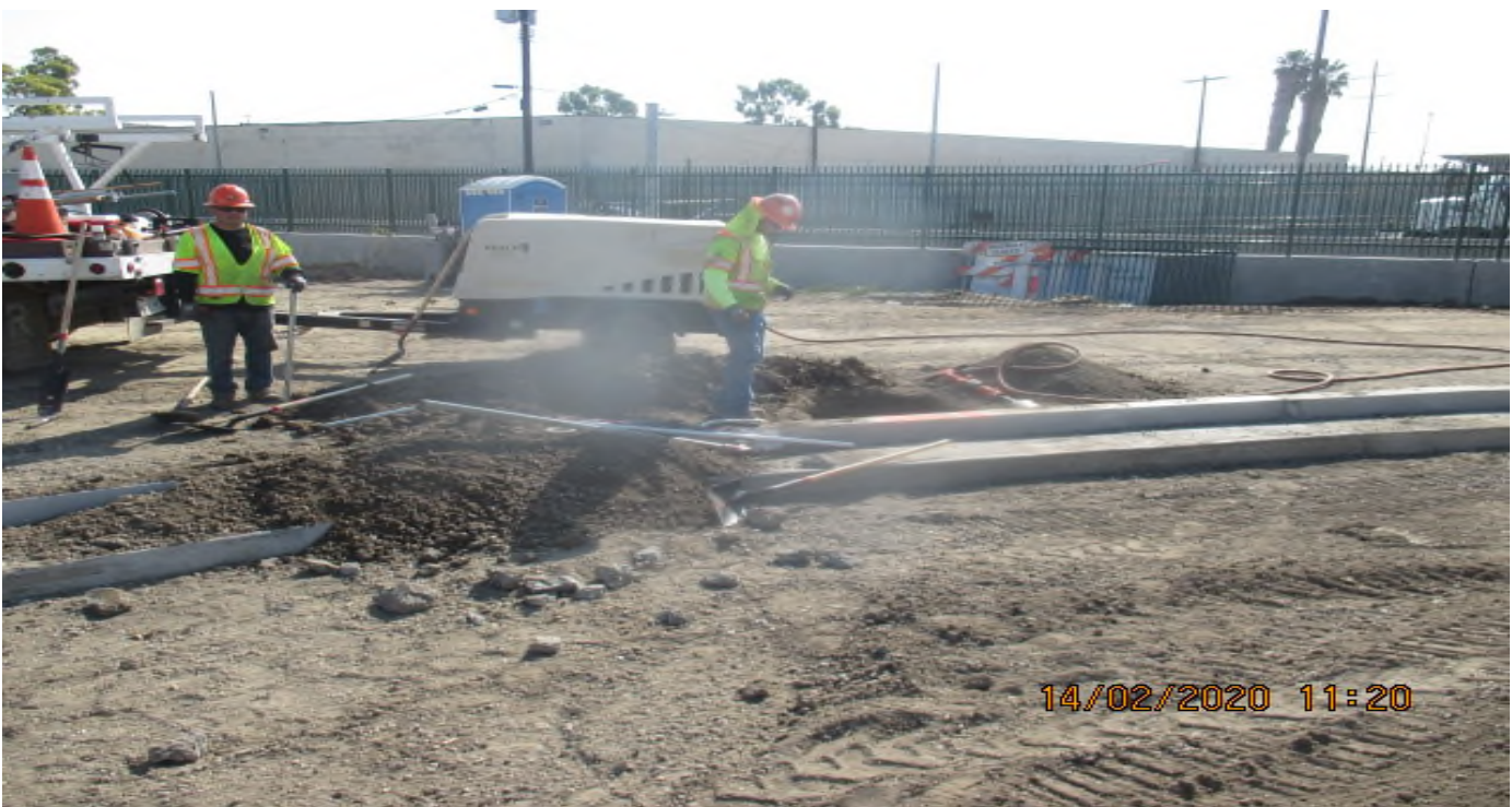
UG3 – Began excavating and installing conduit for street light power on the eastside of the new Cul-de-sac radius at North Victoria Ave. 2/14/20
