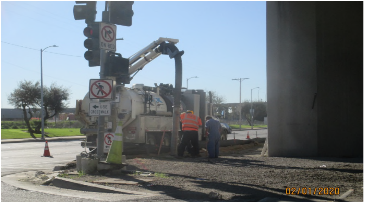
111 STREET – Vacuum truck exposing the gas line at the SW corner of 111th street and Aviation.
