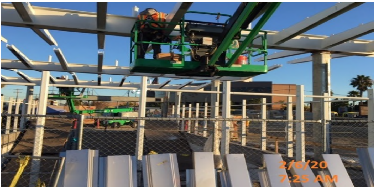
EXPO STATION – Began gutter installation on top of the main entrance canopy structure at the plaza level.
