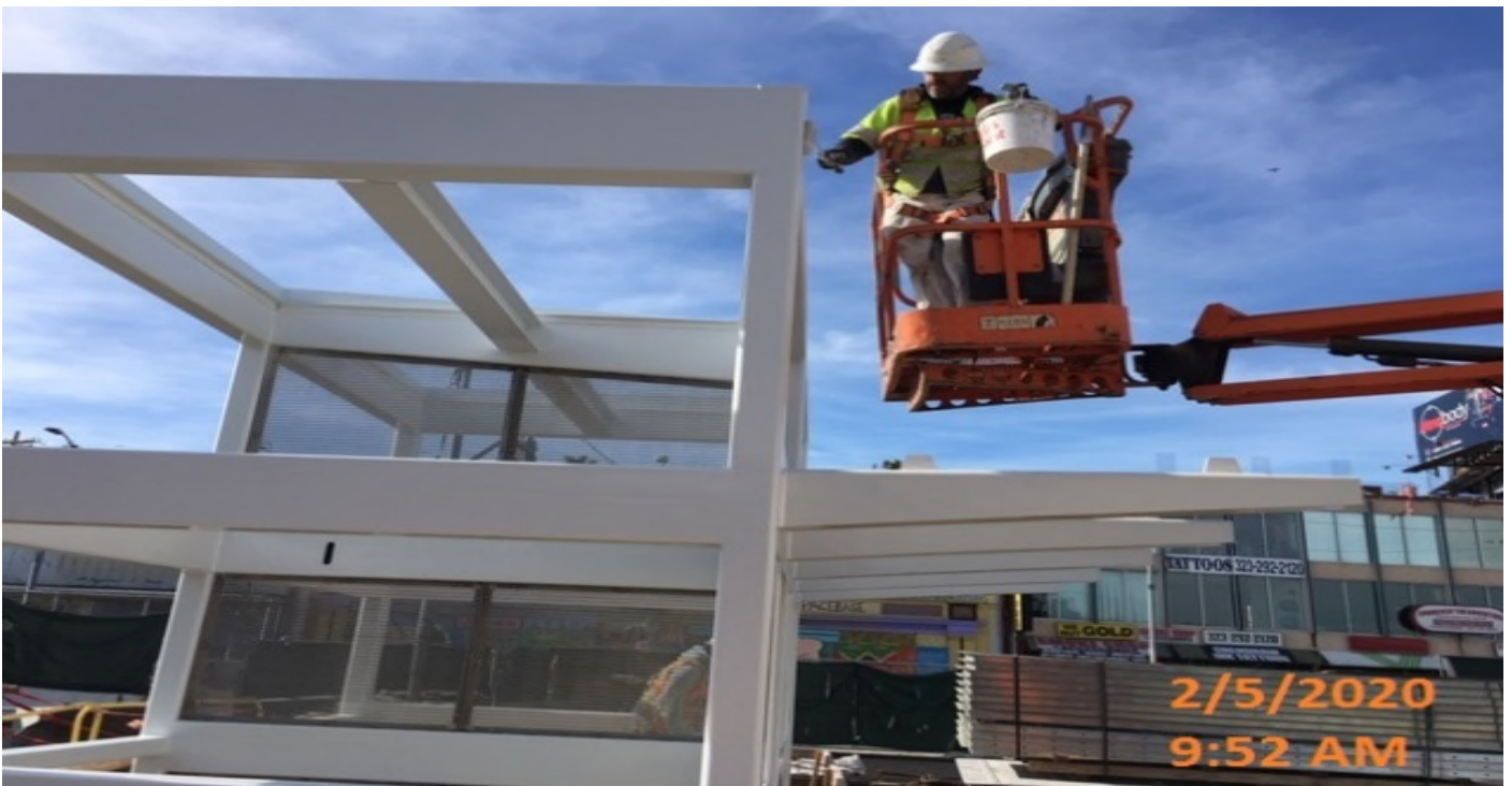
LEIMERT PARK STATION – Applying second coat of finish paint on Elevator structures 1&2 at the plaza level.
