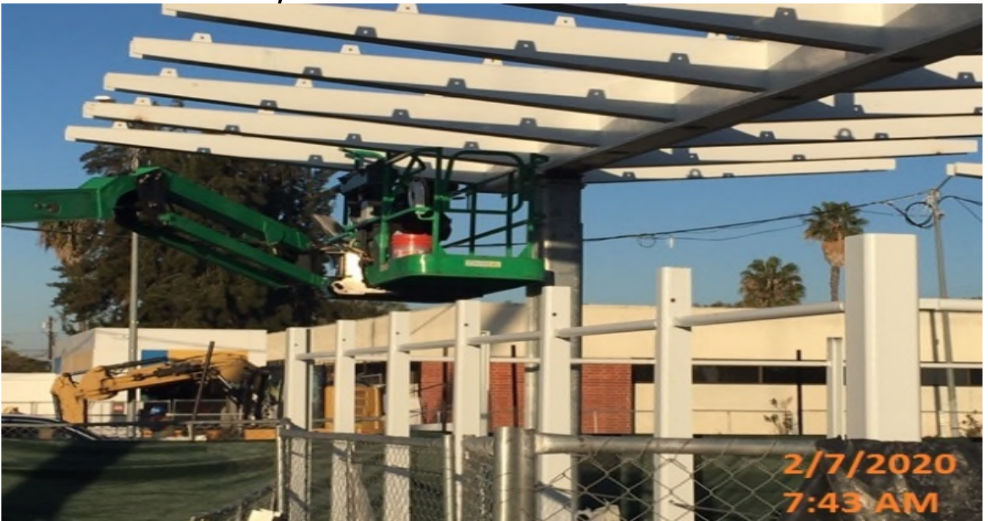
EXPO STATION – Continued gutter installation on top of the main entrance canopy structure at the plaza level.
