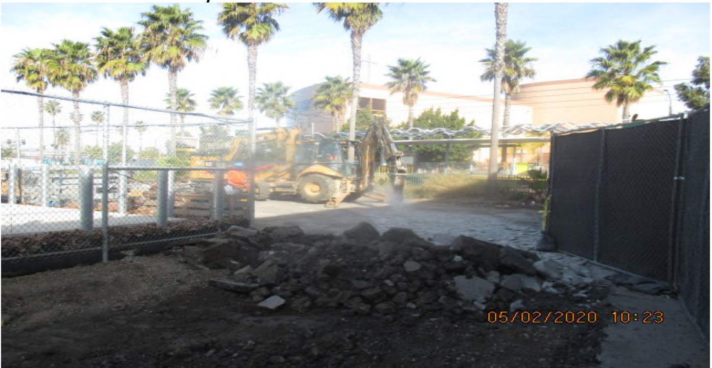
EXPO STATION – Continued demolishing and excavating for the new Cul-de-sac construction on Bronson St. east of the plaza. 2/5/20
