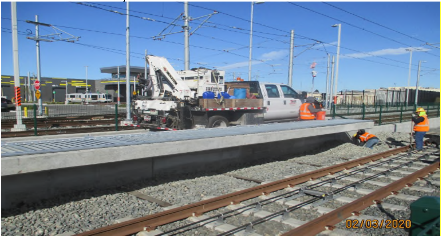
96 th STREET: Layout of the handrail at the 96th Street Station operators platform.
