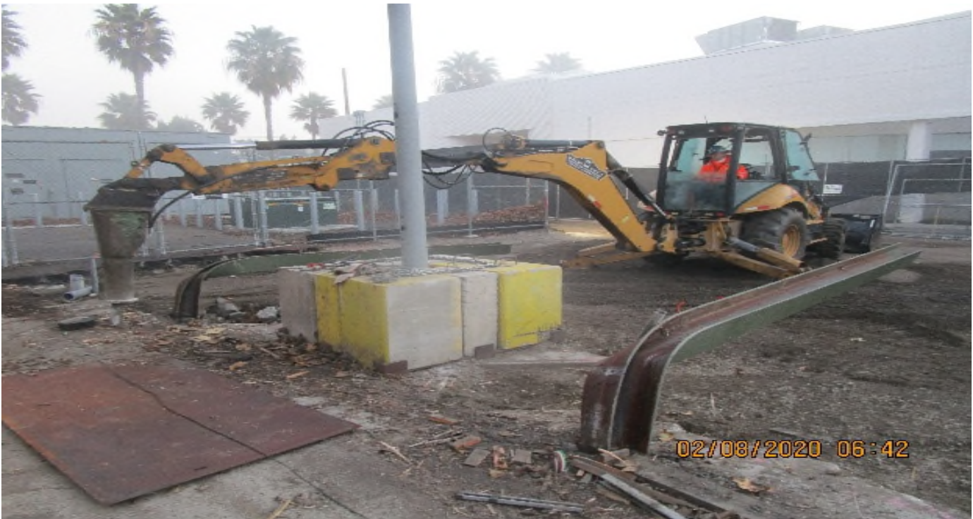
EXPO STATION – Continued demolishing and excavating for the new Cul-de-sac construction on Bronson St. east of the plaza. 2/7/20
