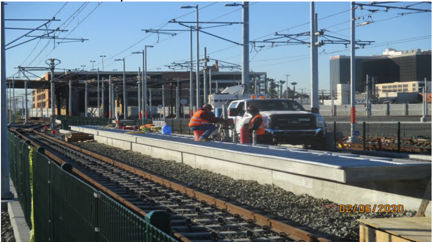
96 th STREET- Core drilling the handrail post holes at the operator's platform.
