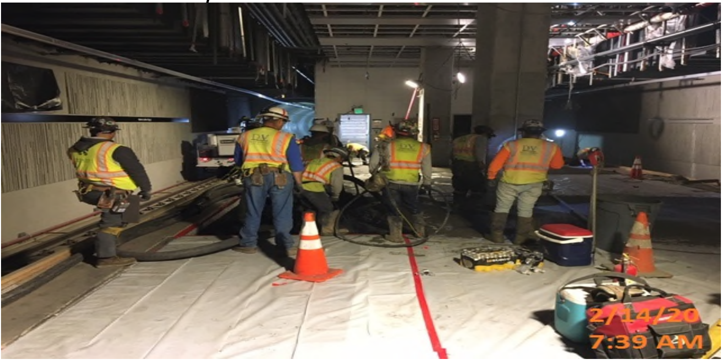
MLK STATION – Began 3rd phase of concrete placement of the architectural topping slab at the platform level.
