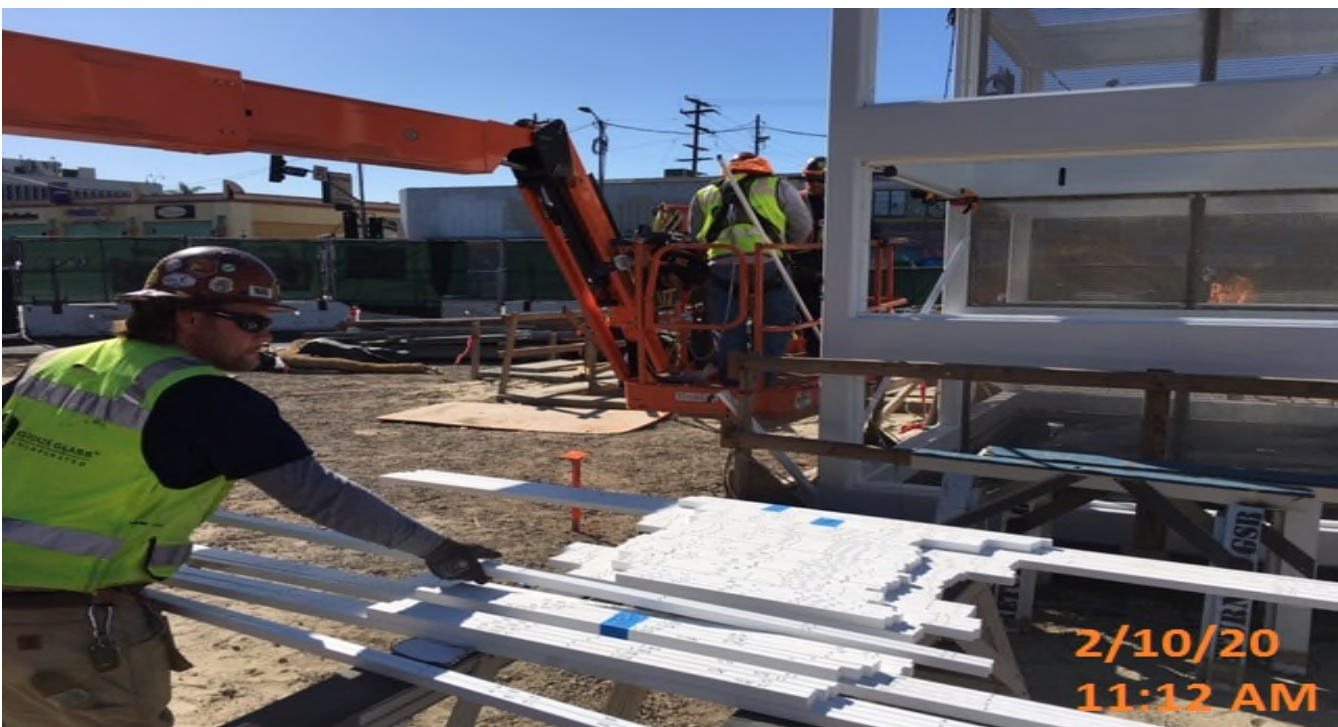
LEIMERT PARK STATION – Installing glass stops for Elevator structures 1&2 at the plaza level.
