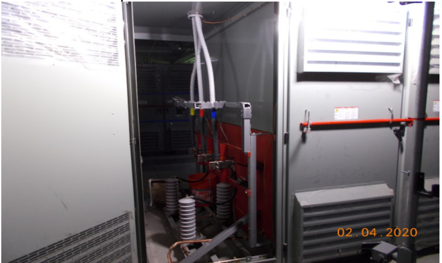
VERNON STA – Faith Electric was finishing securing and landing cables for PX2N
