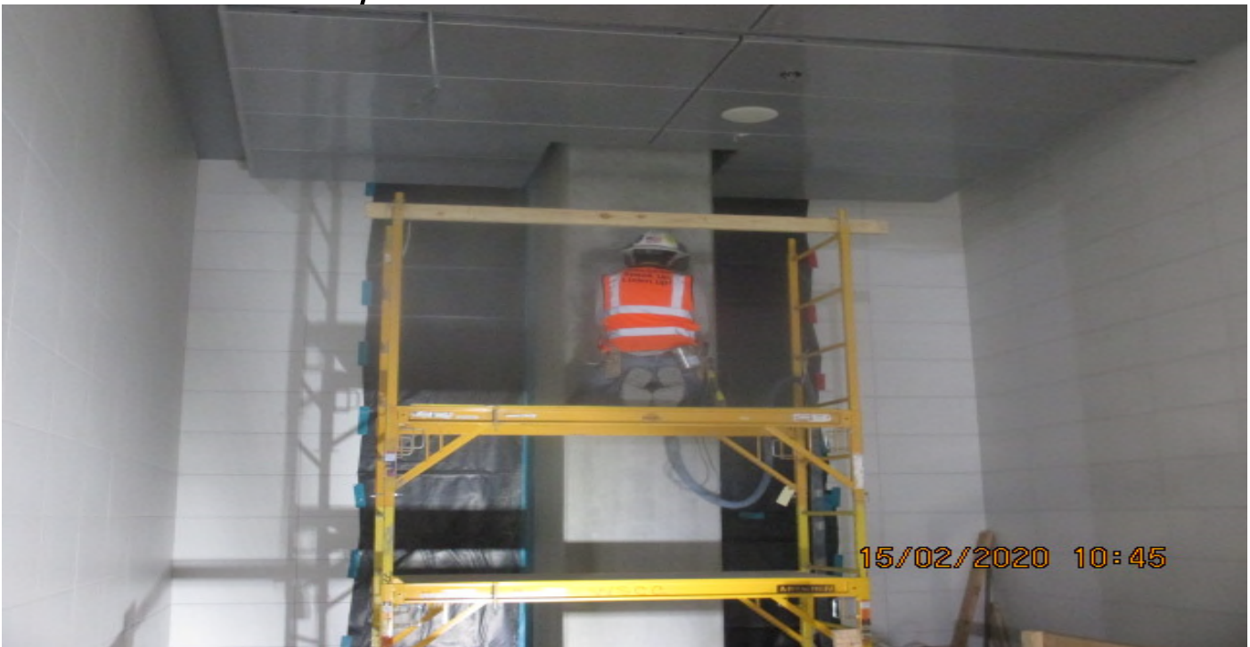
MLK STATION – Continued grinding and smoothing columns in the Free Area of the concourse level. 2/15/20
