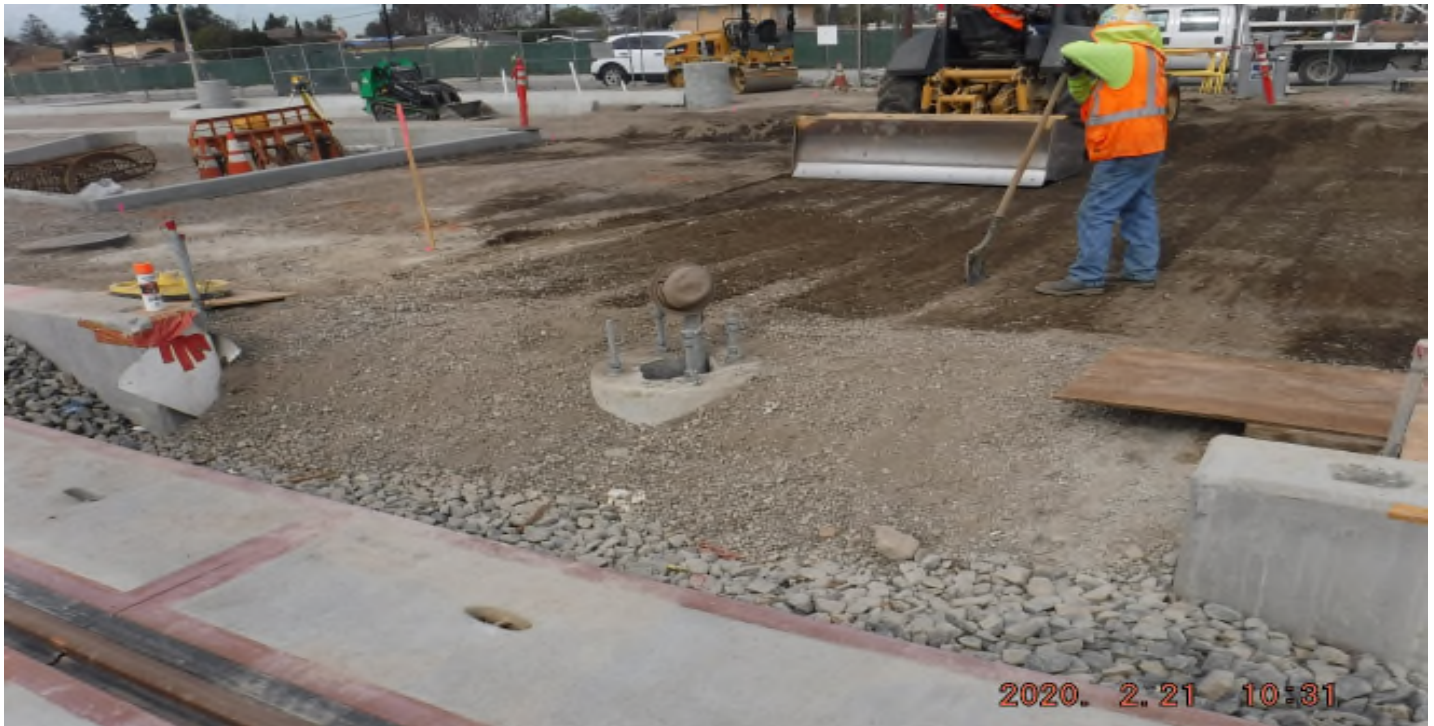
WEST STATION- STA262+74_ lookS_ Gridding next to ped at gr xing_ Sub-ballast migrate in track ballast_ PUNCH LIST
