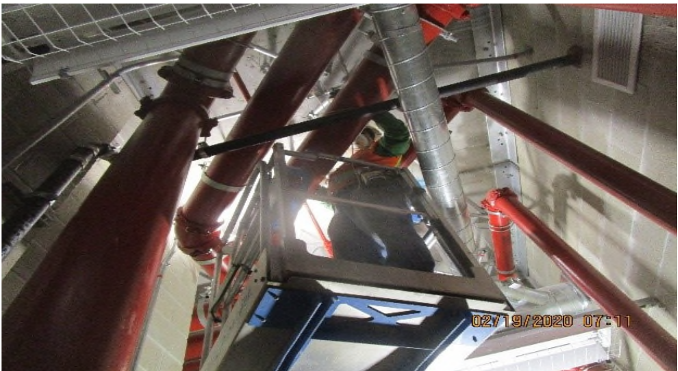
VERNON STA – Sprinkler valve room (S) C116 Overhead Begin pipping 1" GRC to 6"x6"x6" pull box & smoke detector
