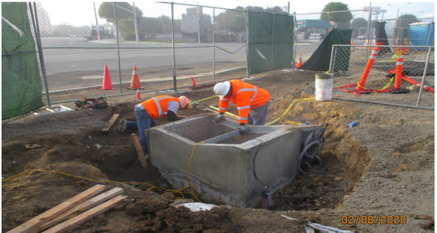
LA BREA – Catch basin concrete finish work at the La Brea Station.
