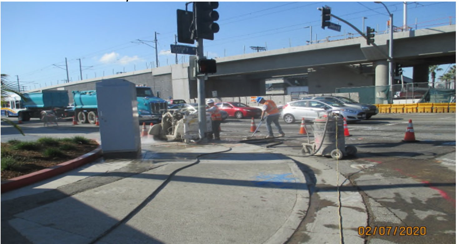
AVIATION/CENTURY- Saw cutting for the demo of the curb & gutter on Aviation & Century.
