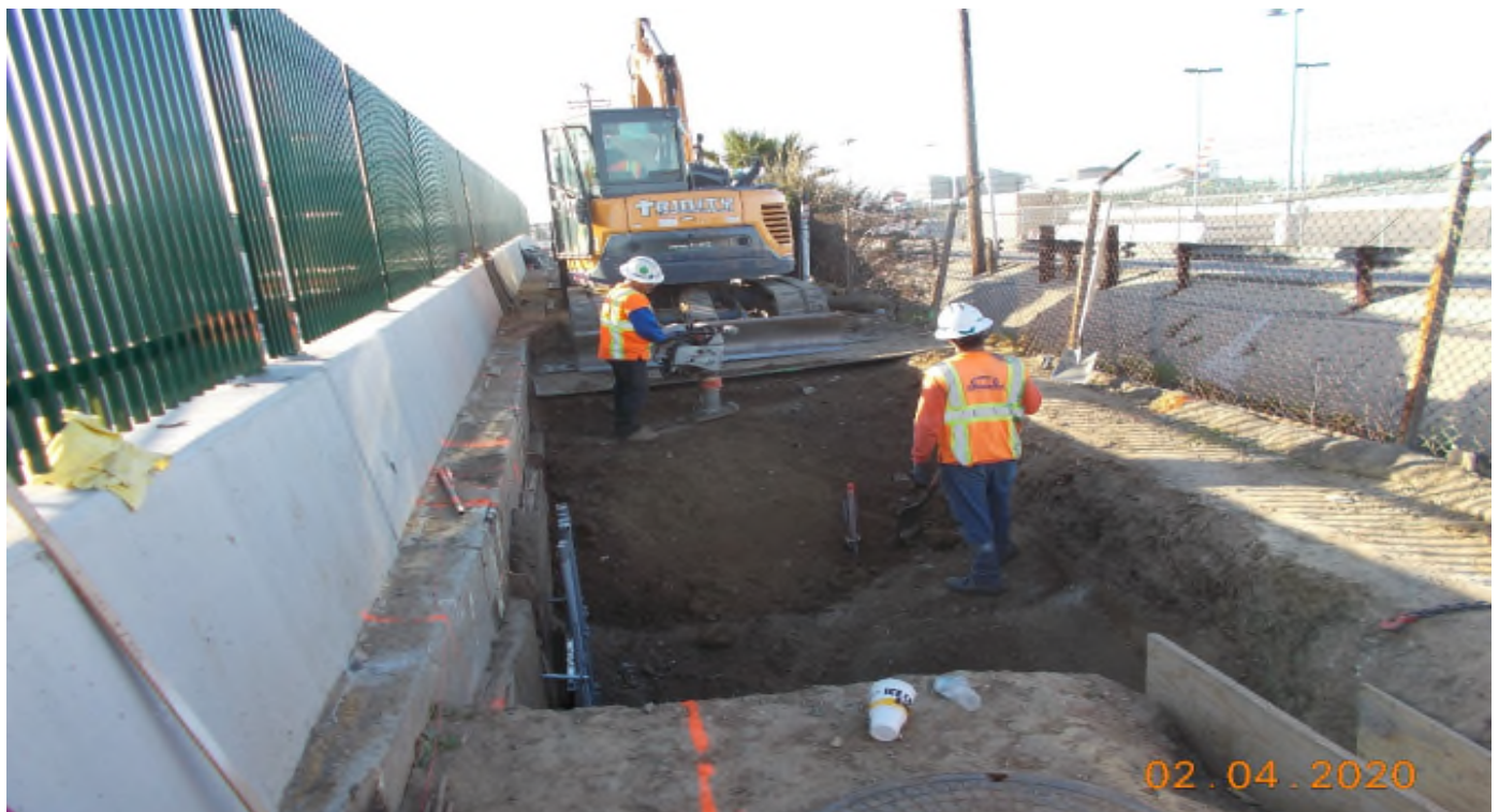
104th St Substation - WA Rasic was backfilling and compacting a power duct bank.
