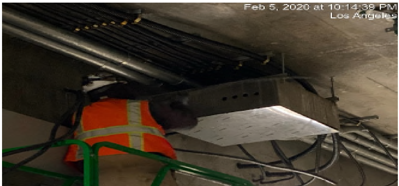
UG-4- Continue wiring and running cable for the booster fans at the southbound tunnel at Sta 377+95.
