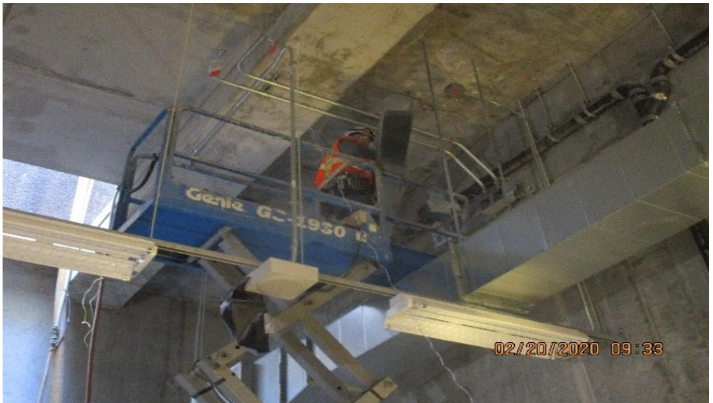
MLK STATION – MLK TPSS Room T109, continued installing drip pans at 4" cast iron concourse level emergency & area drains
