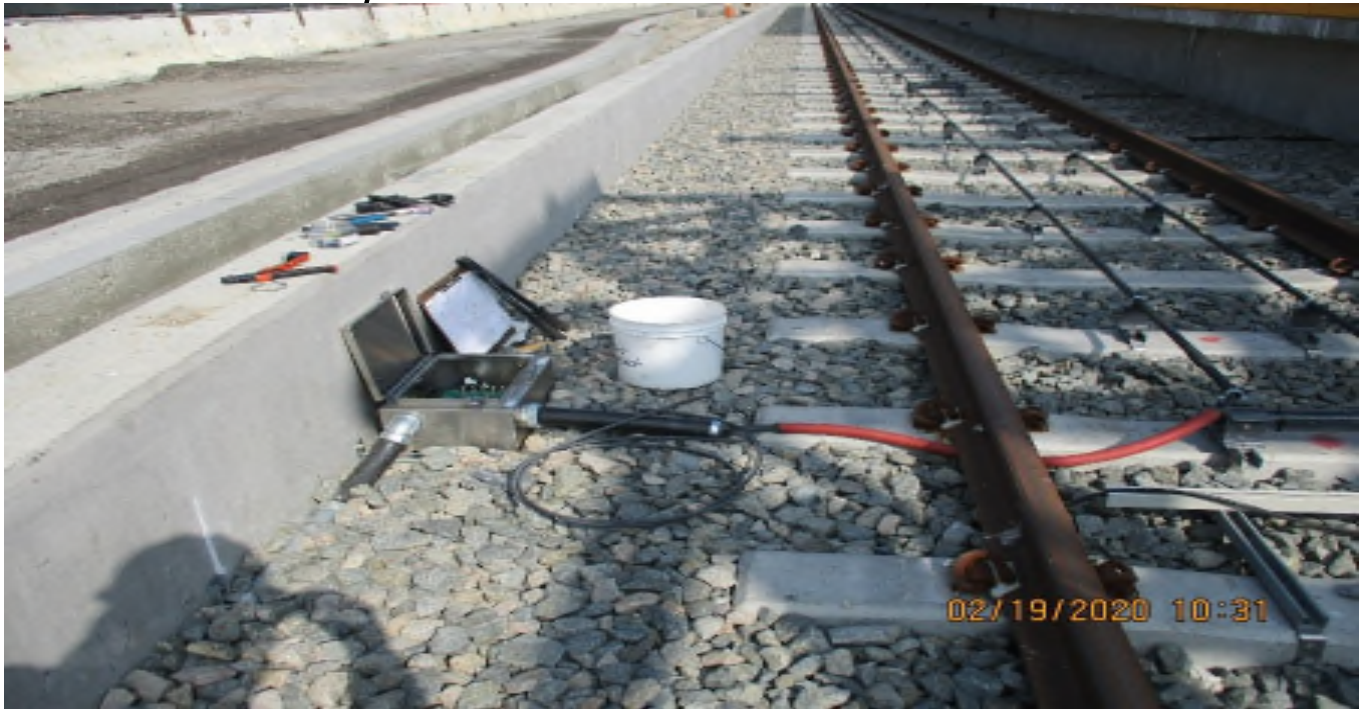
HYDE PARK- LKC Personnel Terminating the Cables for Coupling Unit 3CU320, Looking North
