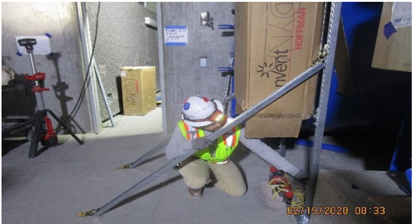
MLK STATION – Emergency Fan room (S) EVF pull box support rack kickers encroaching into path of travel means of egress.
