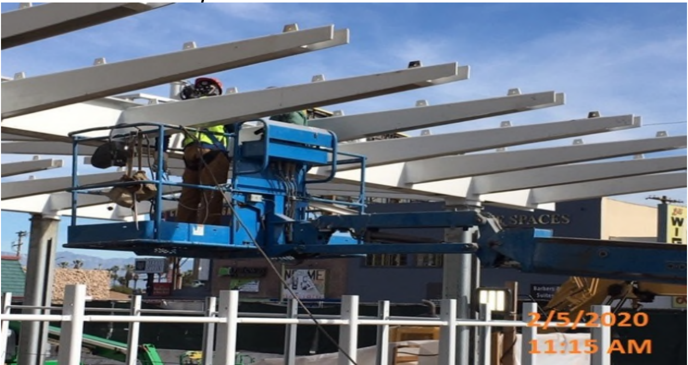
MLK STATION – Began catwalk installation and continued gutter installation on top of the main entrance canopy structure at the plaza level.
