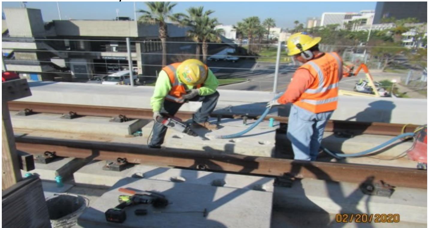
AVIATION/CENTURY- WSCC using E-hammer to chip out inserts holes on Century, Aviation bridge SB #3 track STA 66+09 (looking west).
