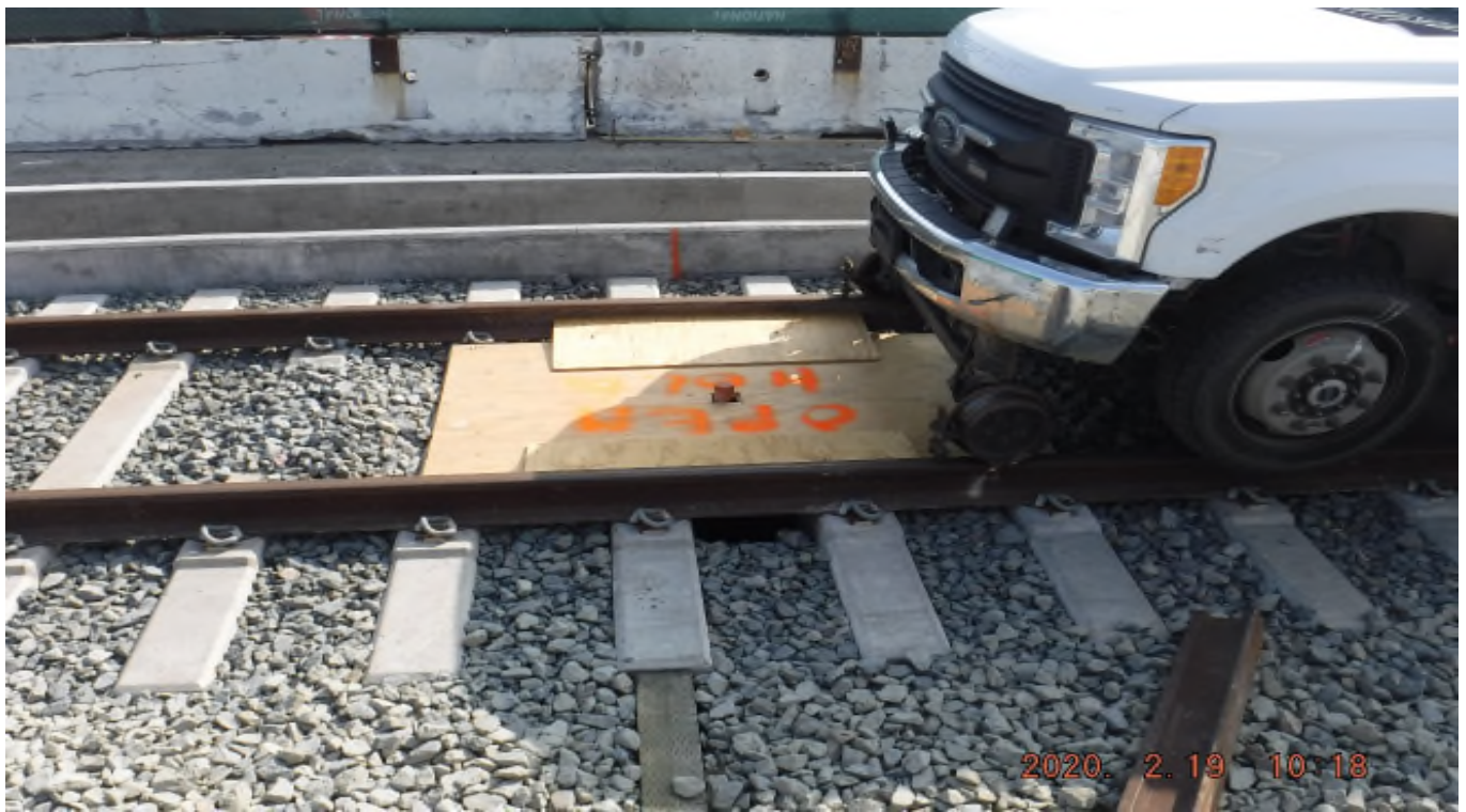
SLAUSON STA- STA322+66_ Looking East_ Disturbed track structure_ PUNCH LIST.
