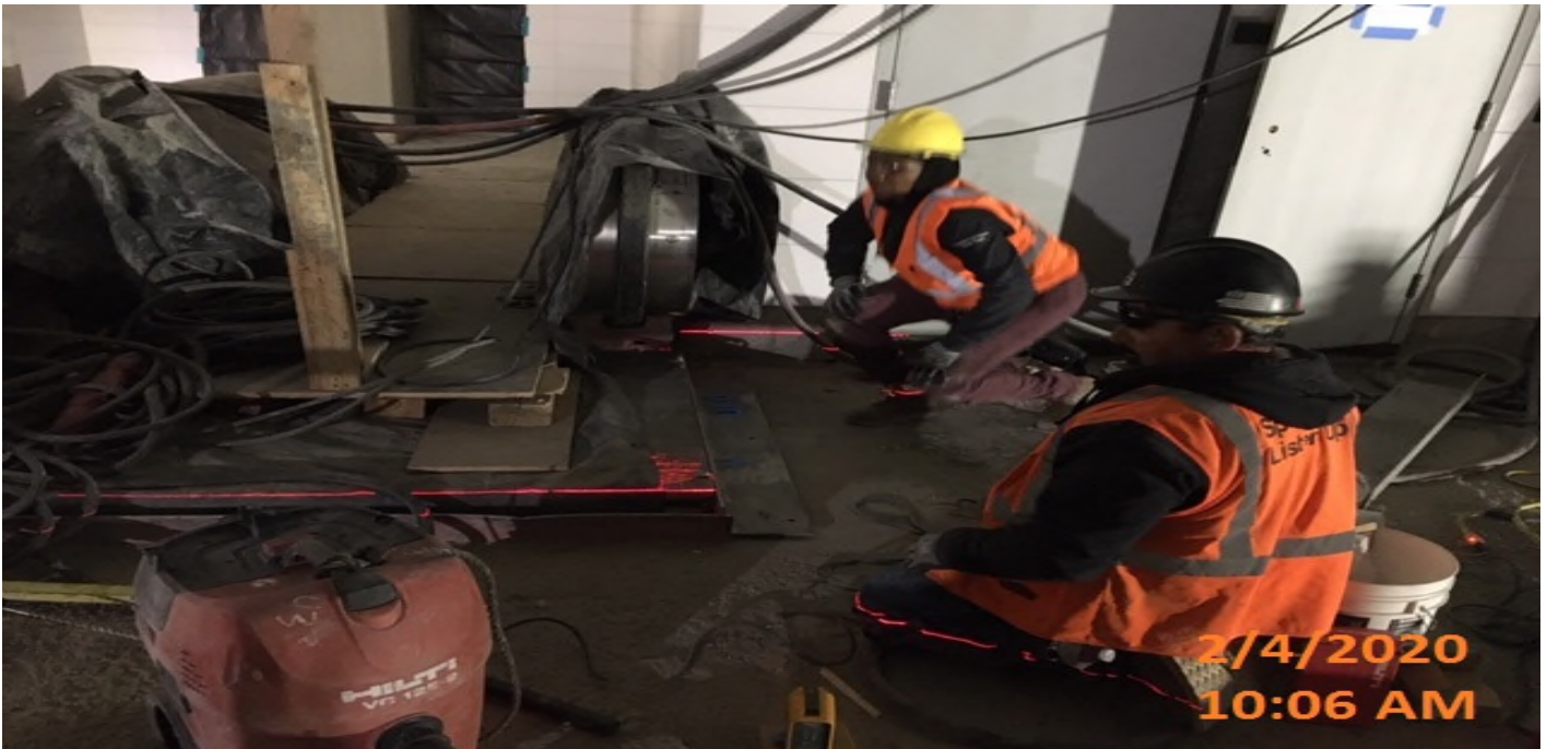
MLK STATION – Installing bent plates at the landing of Escalator #4 on the concourse level.
