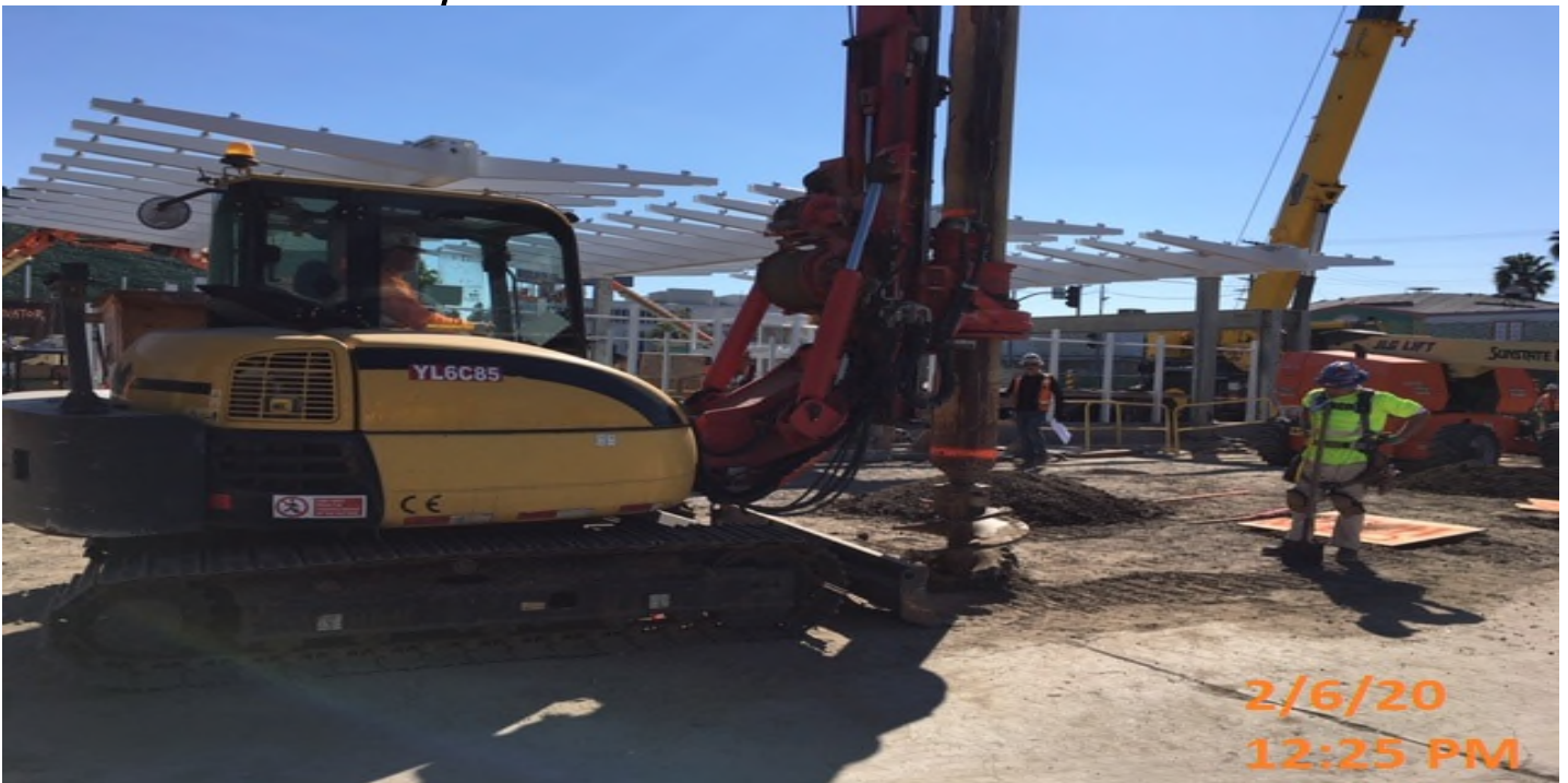
LEIMERT PARK STATION – Drilling for the installation of the luminaire light posts at the plaza level.
