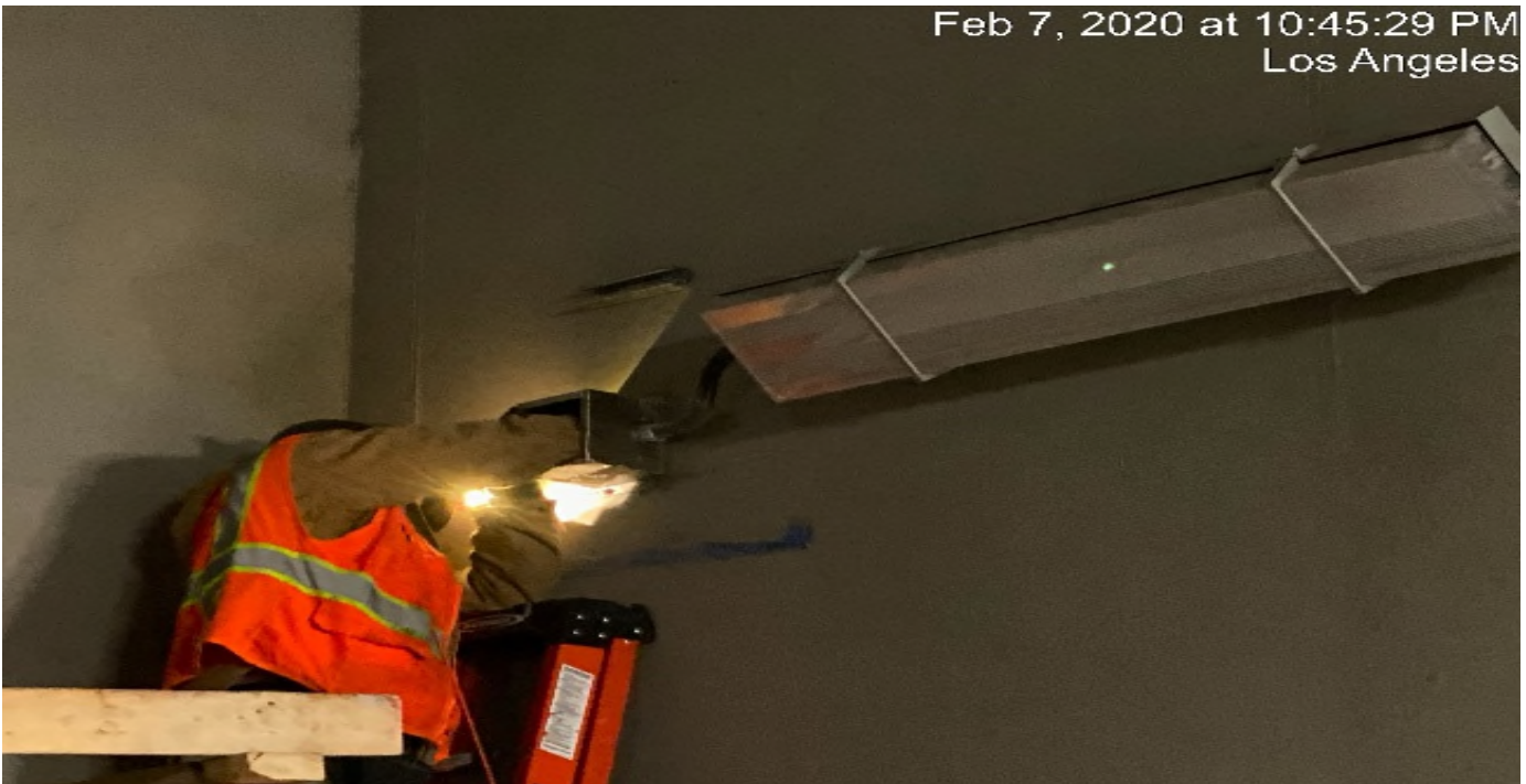
UG-4- Continue pulling wire for the emergency lighting at the south end portal entrance.
