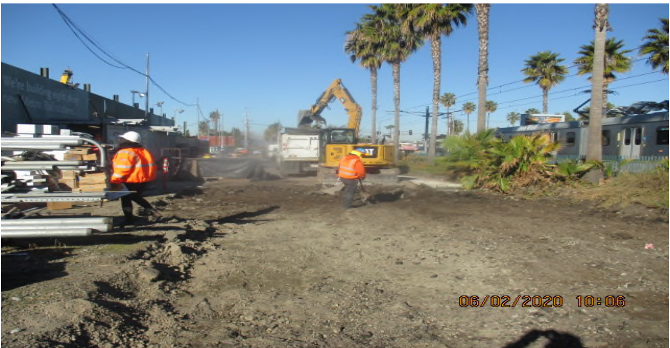
EXPO STATION – Continued demolishing and excavating for the new Cul-de-sac construction on Bronson St. east of the plaza. 2/6/20
