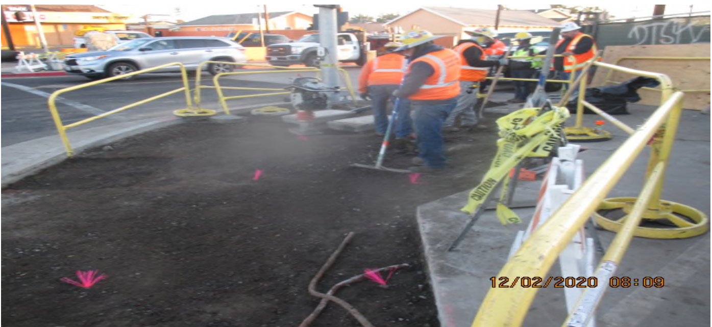
UG3 – Began backfilling/compacting for new installation and concrete placement of sidewalk and ADA ramp on the southeast corner of 67th St and Crenshaw Blvd. 2/12/20
