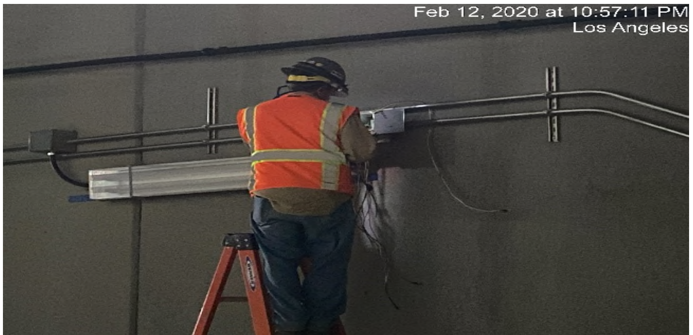
UG3 – Continue pulling wire for the emergency lighting at the south end portal entrance.
