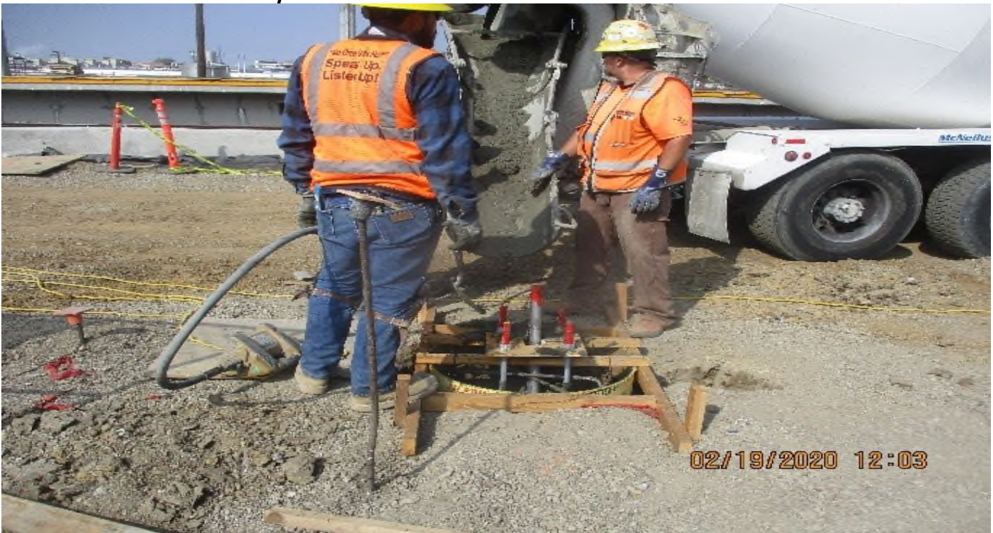
LA BREA - WSCC Placing conc for light foundations at La Brea park and Ride.
