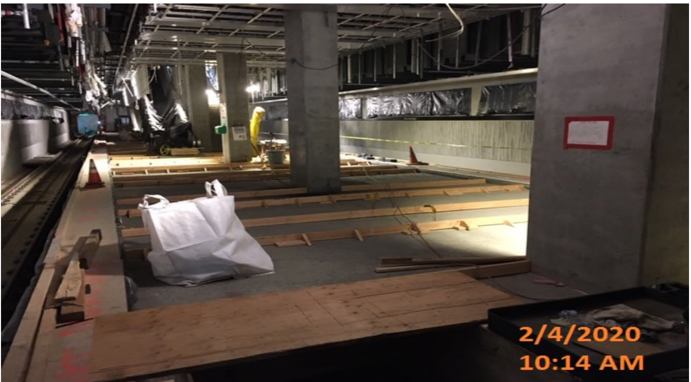
MLK STATION – Began formwork for the architectural topping slab at the platform level.
