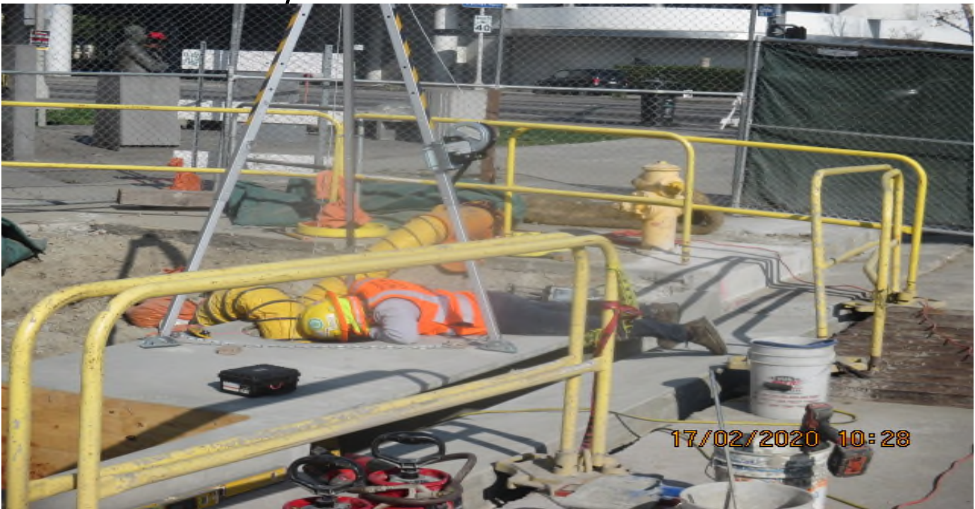
MLK STATION – Prepping valve pit access hatch formwork for concrete placement at the plaza level.
