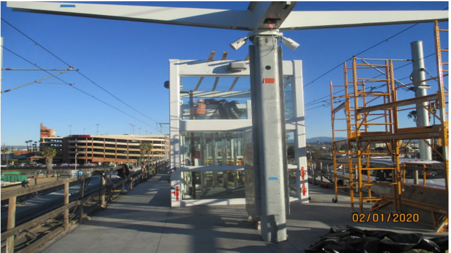
AVIATION/CENTURY- Removal of the rain cover and wood at the Aviation Station elevators.
