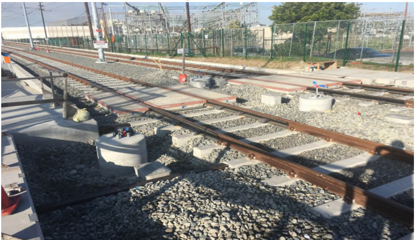
HINDRY AVE- STA131+40_ looking South_ Track structure disturbed _PUNCH LIST.
