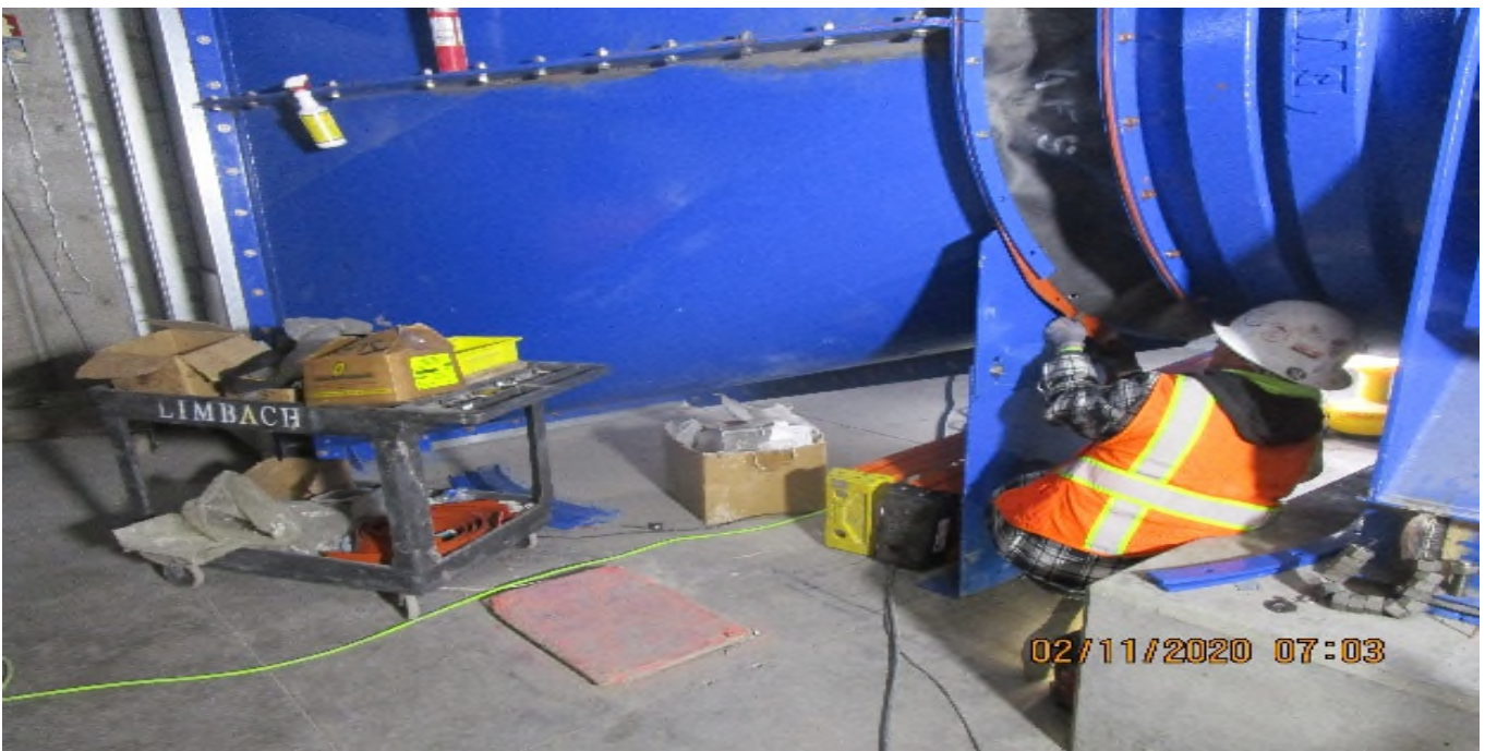
LEIMERT PARK STATION – Continued installing silicone gaskets and roughing in flex connectors to EVF-6-302 in the North Fan Room C – 126 Fan Rooms of the concourse level.
