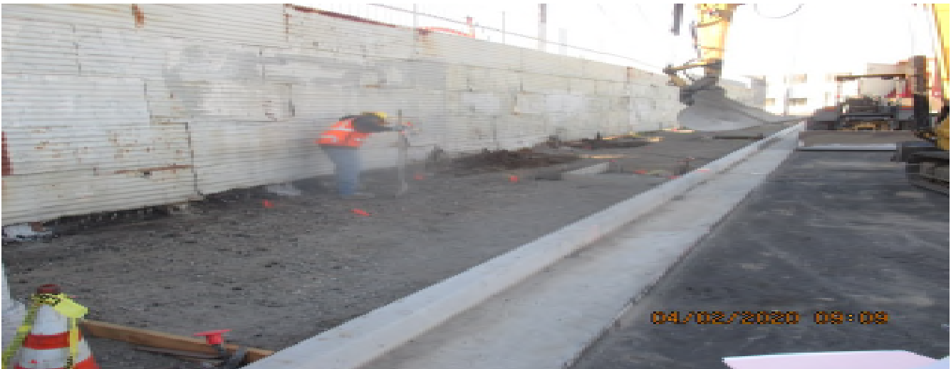
UG3 – Completing final excavation of eastbound “New Road” sidewalk in preparation for curb/gutter installation and concrete placement. 2/4/20
