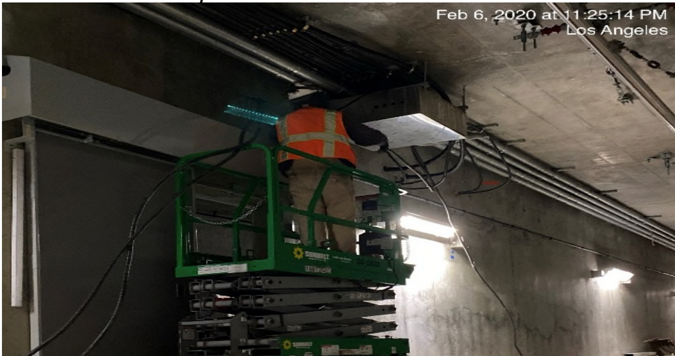
UG-4- Continue wiring and running cable for the booster fans at the southbound tunnel at Sta 377+95.
