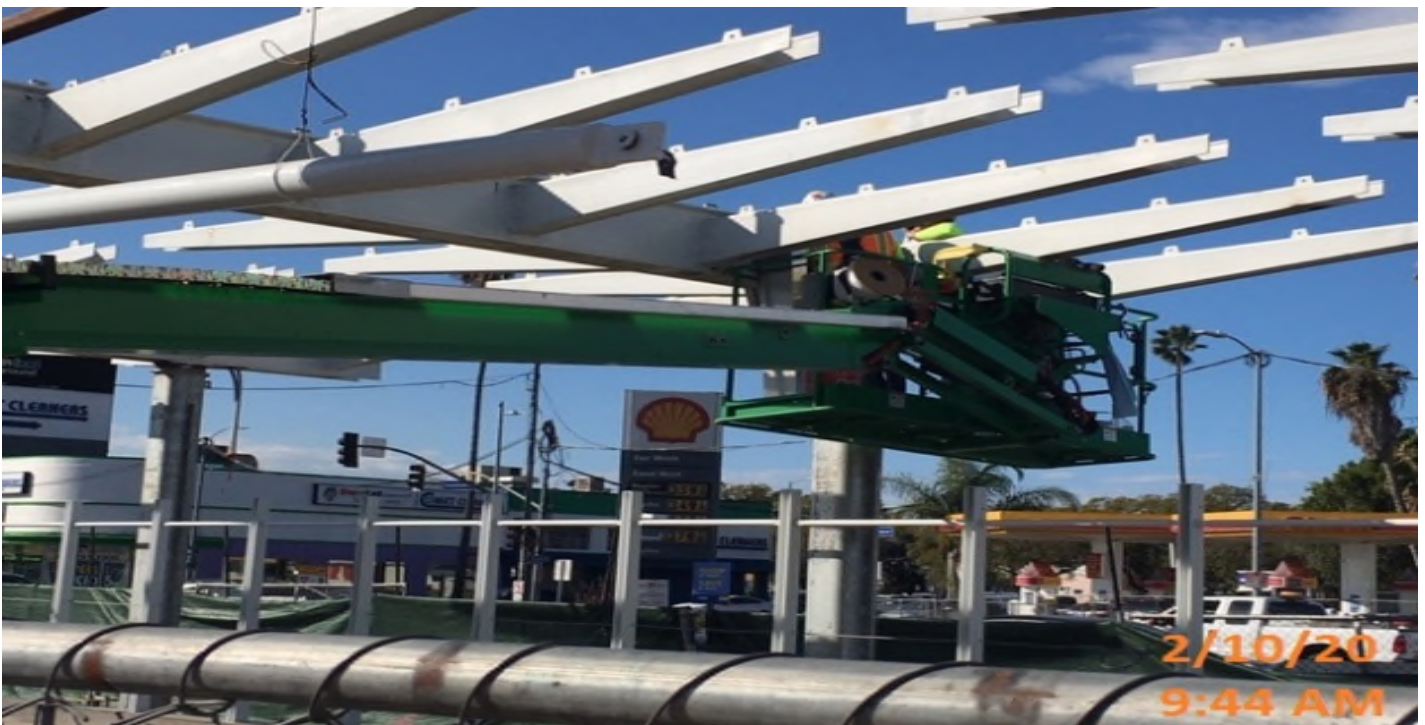
EXPO STATION – Continued gutter installation on top of the main entrance canopy structure at the plaza level.
