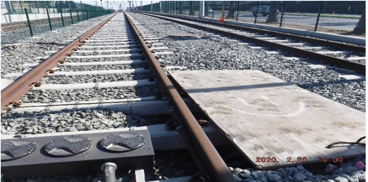
HIGH STREET- STA 249+50 SB looking north – disturbed track structure @ S461, S462 (Centinela – High) – PUNCH LIST
