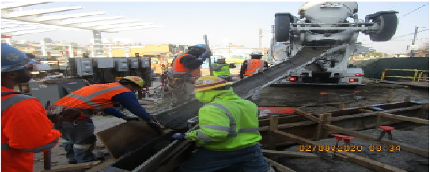
LEIMERT PARK STATION – Continued placing concrete on both the north and south section planter walls at the plaza level.
