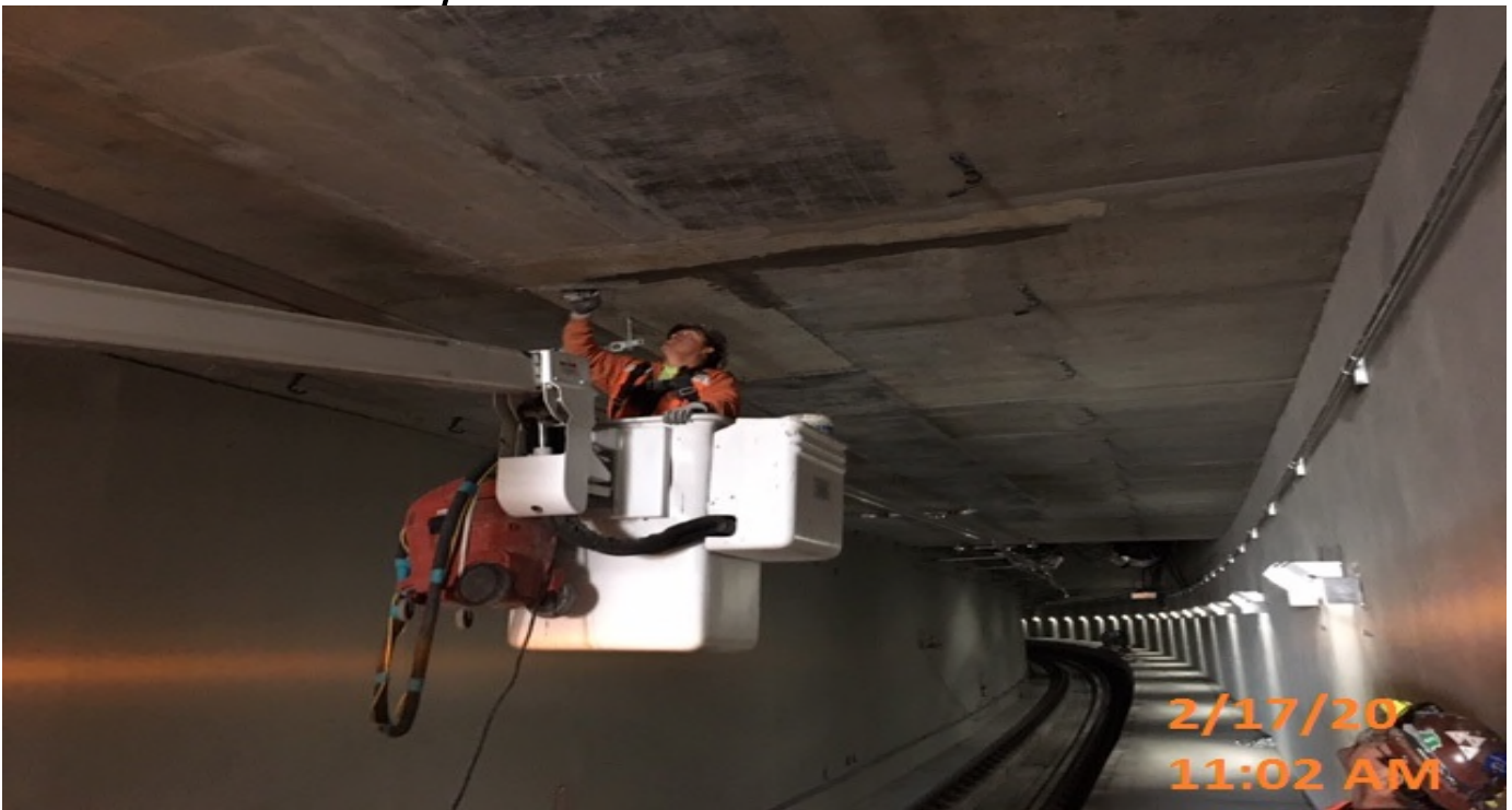
UG-4- Continue sack and patch of ceiling along the southbound tunnel from Sta 372+00 – 377+26.
