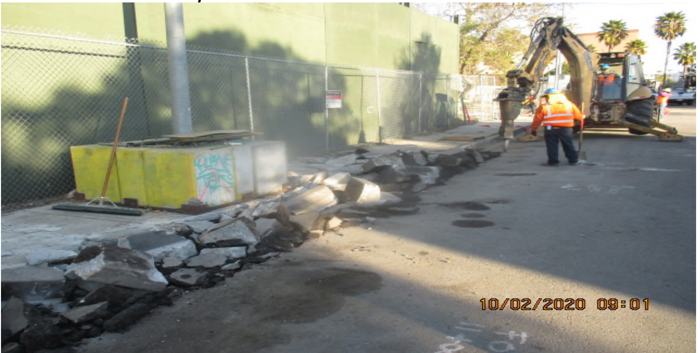
EXPO STATION – Demolishing and excavating curb/gutter for the new Cul-de-sac construction on Bronson St. east of the plaza. 2/10/20
