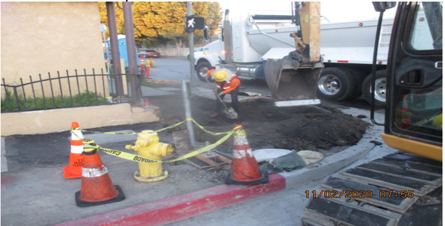
UG3 – Excavating and removing temporary AC for new installation and concrete placement of sidewalk and ADA ramp on the southwest corner 63rd St and Crenshaw Blvd. 2/11/20
