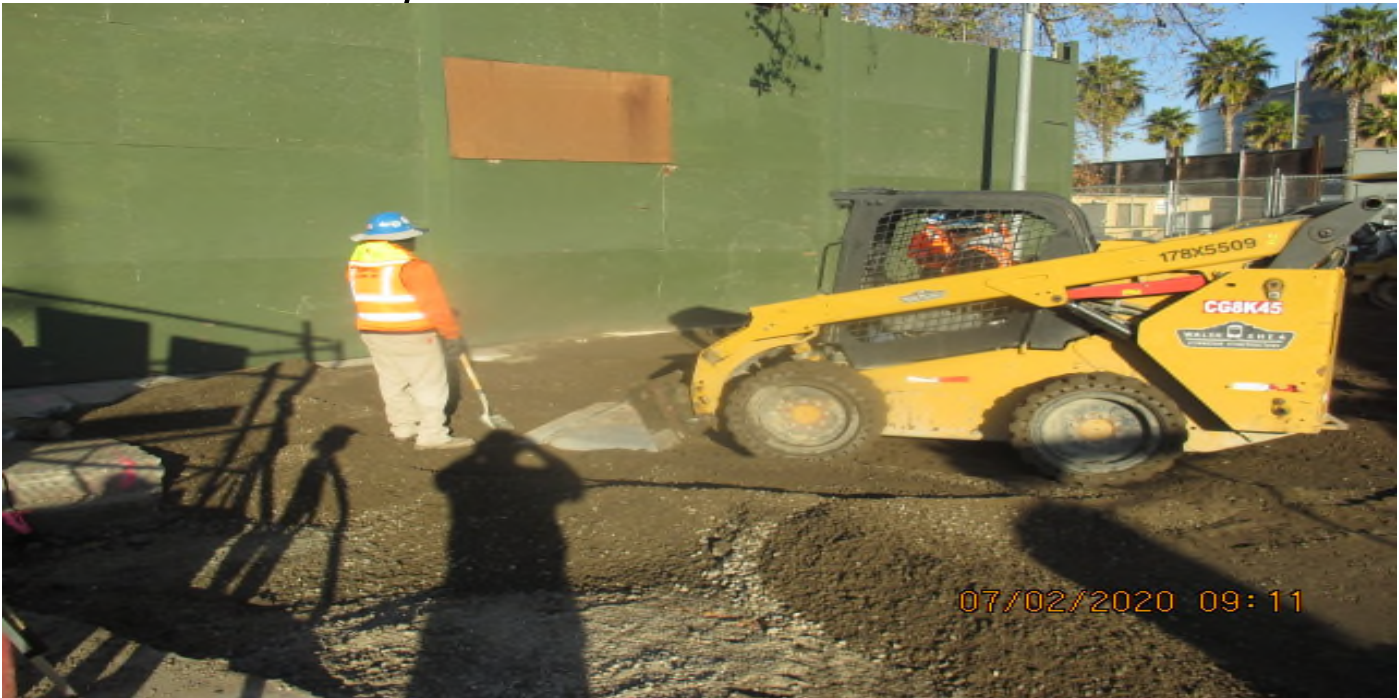
EXPO STATION – Continued excavation/backfill for the new Cul-de-sac construction on Bronson St. east of the plaza. 2/7/20
