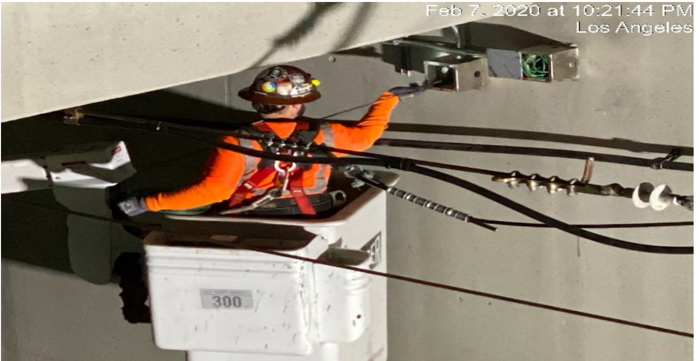
UG3 – Continue pulling wire for the emergency lighting at the south end portal entrance.
