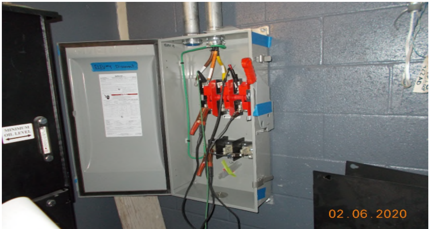
VERNON STA – NETE was megger testing elevator disconnects.
