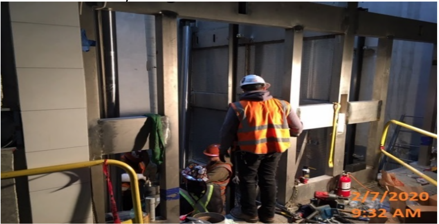
MLK STATION – Continued jack installation inside Elevator hoist way/pits 1&2 at the concourse level.
