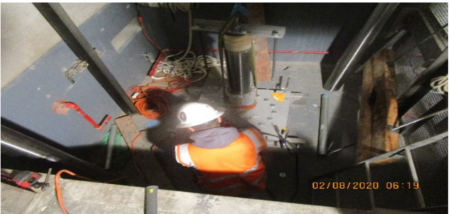
MLK STATION – Continued jack installation inside Elevator hoist way/pit 2 at the concourse level.
