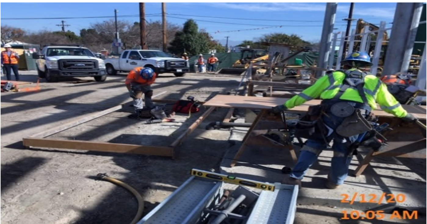
LEIMERT PARK STATION – Continue building formwork for the north emergency shaft ventilation grate and exit hatches at the plaza level.
