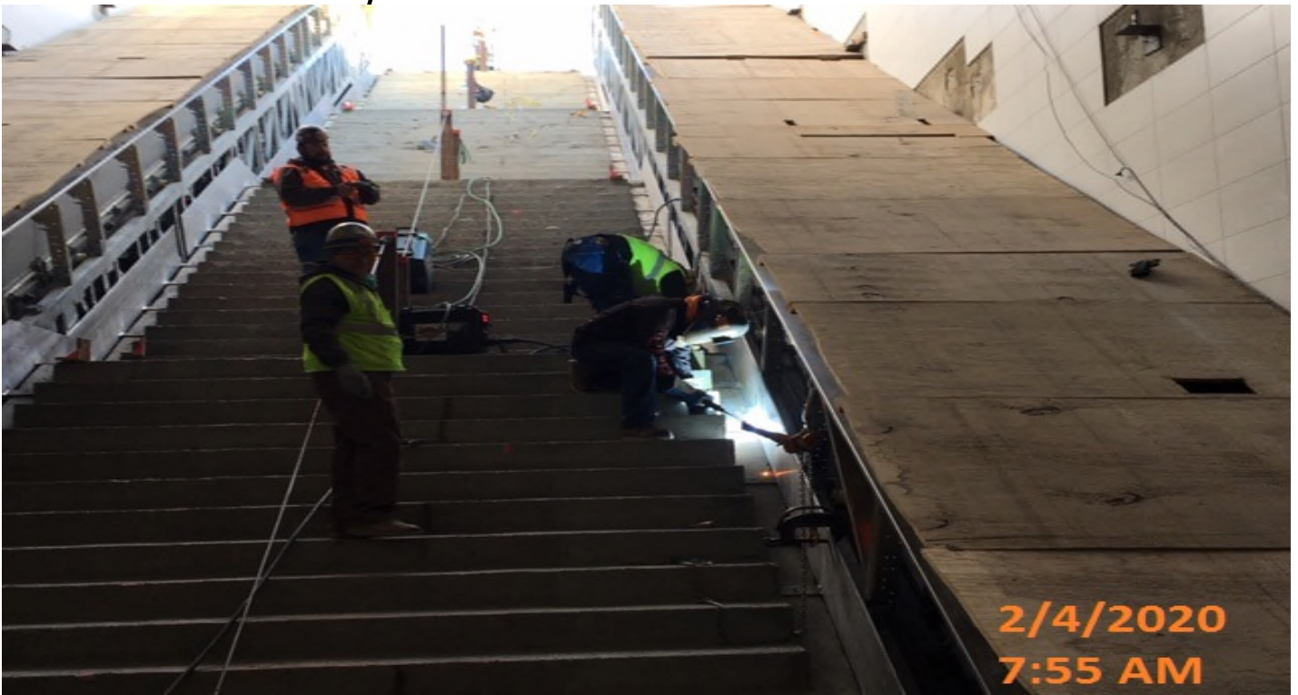
EXPO STATION – Continued installing edge plates for Escalator 1&2 at the main staircase landing of the plaza level.
