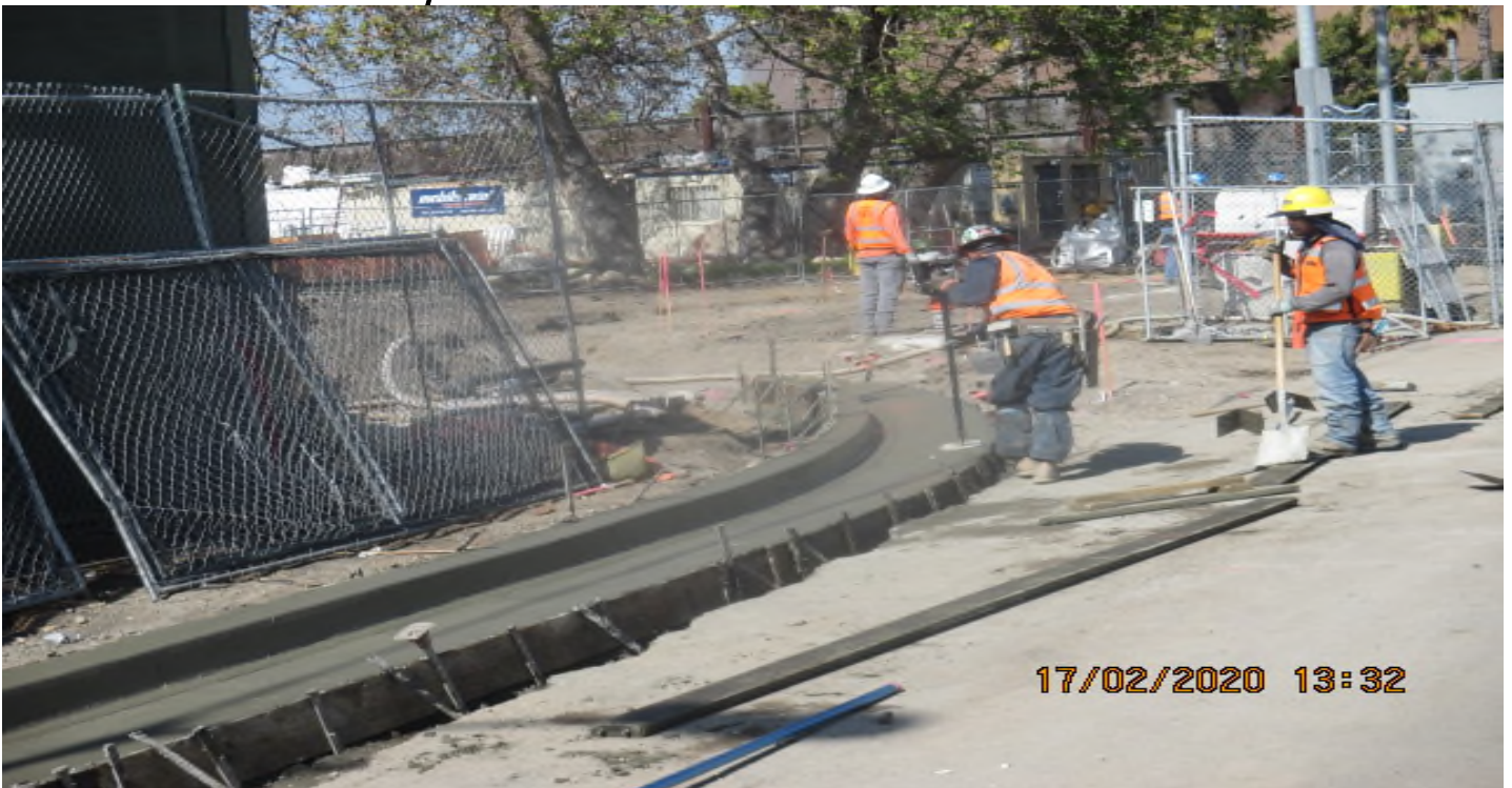
EXPO STATION – Began curb/gutter formwork and placing concrete for new Cul-de-sac radius on Bronson St. east of the plaza. 2/17/20
