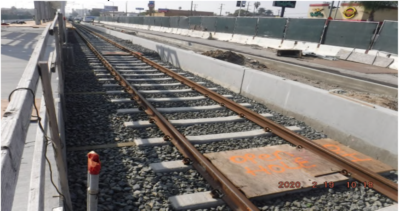
SLAUSON STA - STA322+63_ Looking South_ Disturbed track structure_ PUNCH LIST
