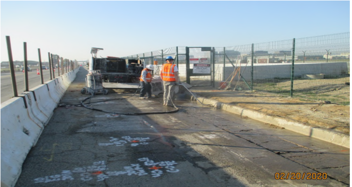
UG 1- Saw cutting the curb at UG-1 to make way for the new driveways on Aviation.
