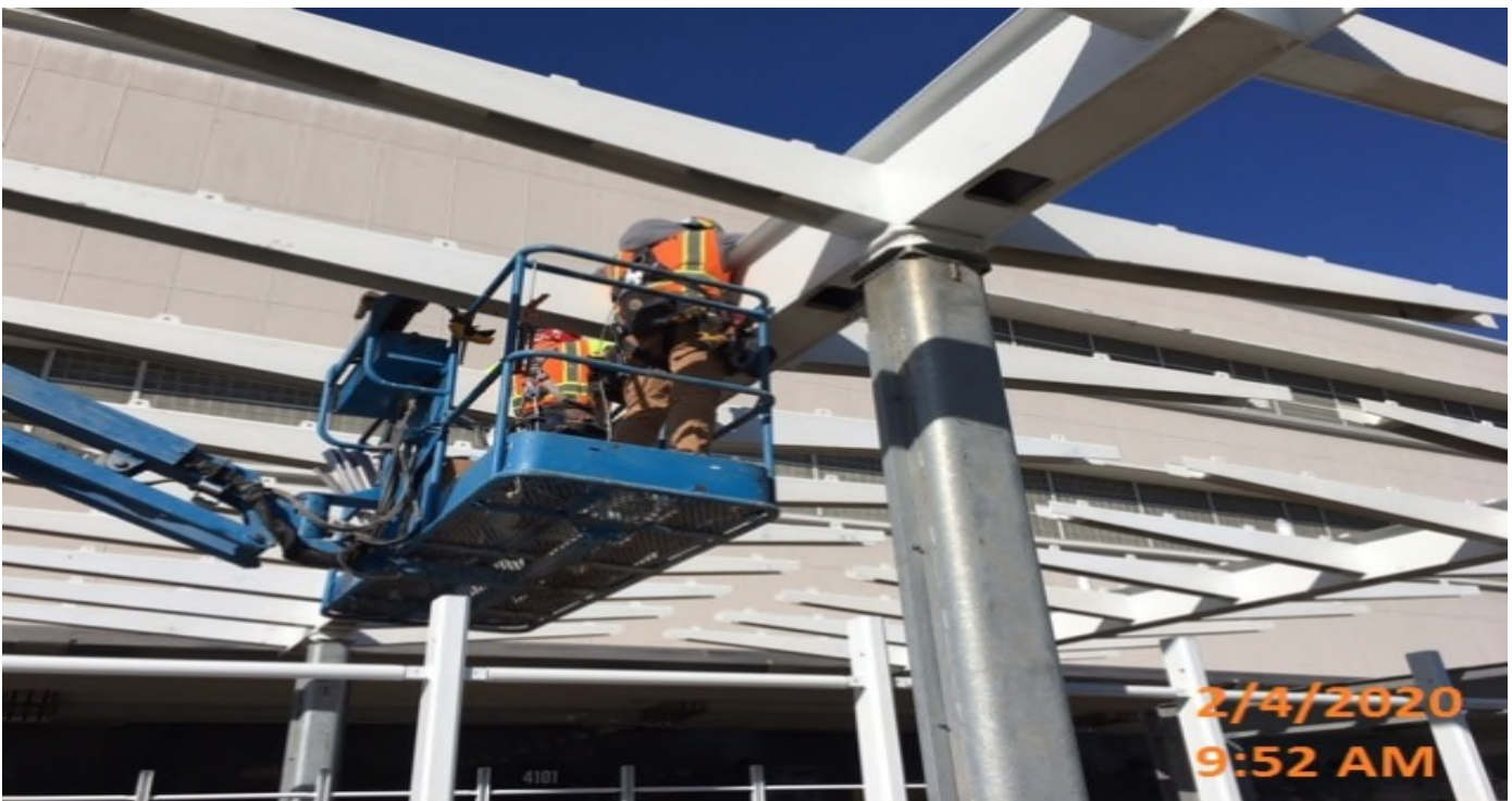
MLK STATION – Began gutter installation on top of the main entrance canopy structure at the plaza level.
