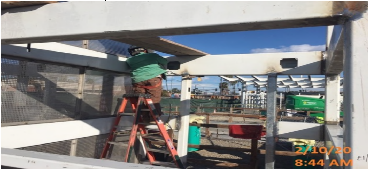
EXPO STATION – Continued grinding welds on HSS member frames of Elevator structures 1&2 at the plaza level.
