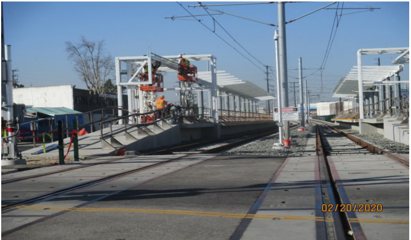
HINDRY AVE- Metal stud installation at the Hindry NB platform. Facing west.
