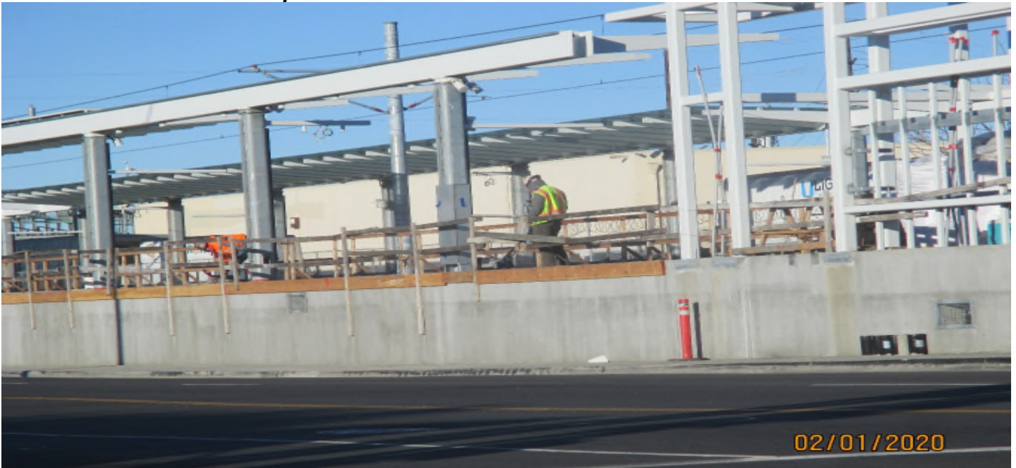
HINDRY AVE- Saw cutting expansion joints and buffing the topping slab at the NB platform.
