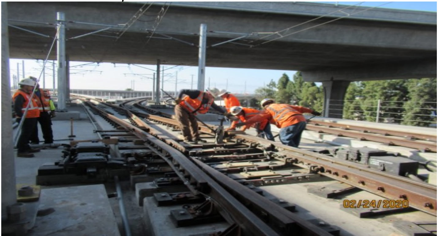
GREENLINE UNDERPASS- HCC working on MPF at GL Wye raising rails for WSCC to work on concrete slab elevation.
