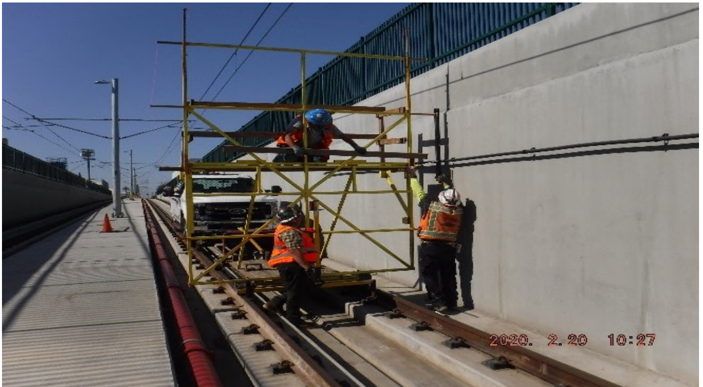
UG3 – STA 278+80 SB looking south – checking VDC clearance UG3 south ramp (Victoria)
