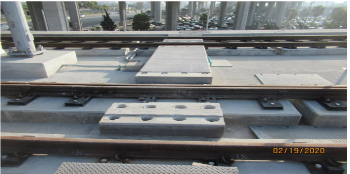
GREENLINE UNDERPASS- East leg of Wye crossing plates incomplete install.
