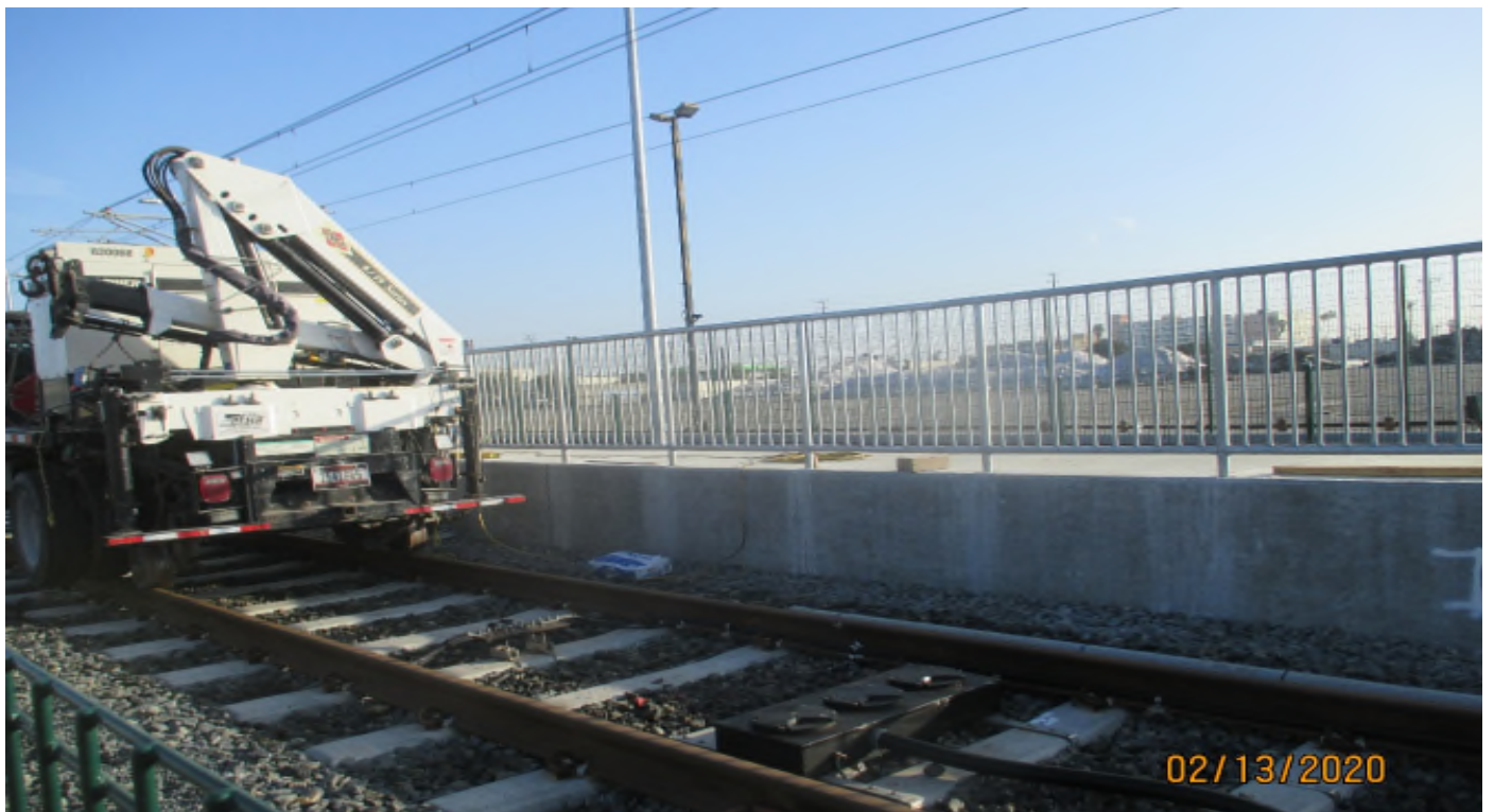
96 th STREET- Grouting the handrail posts for the 96th Street Station operator's platform.
