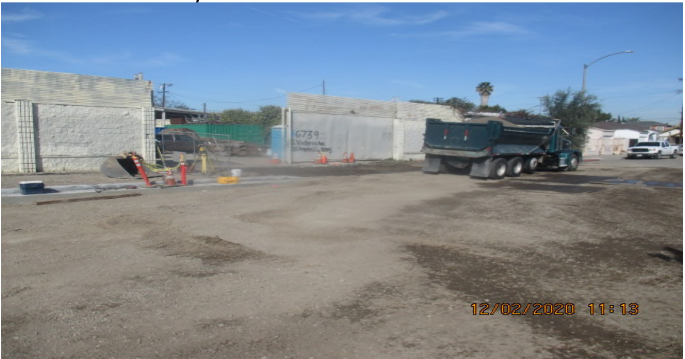
UG3 – Continued excavation/compaction of the new Cul-de-sac in preparation for curb/gutter installation and concrete placement at North Victoria Ave. 2/12/20
