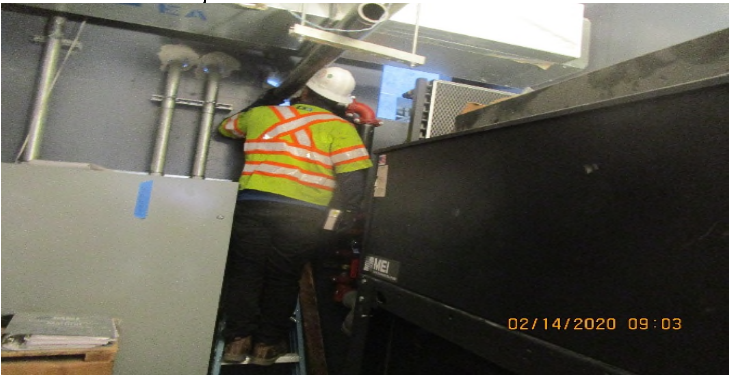
MLK STATION – Continued 3” hydraulic pipe line installation for Elevator 1 at the Machine Room C – 116 of the concourse level.
