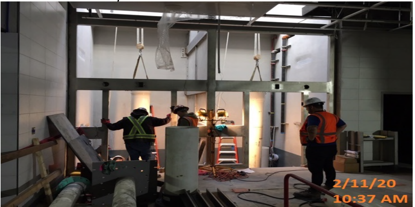
LEIMERT PARK STATION – Continue installing 15” PVC into HDPE sleeve and began starter rails for Elevator hoist way/pit 1&2 at the concourse level.
