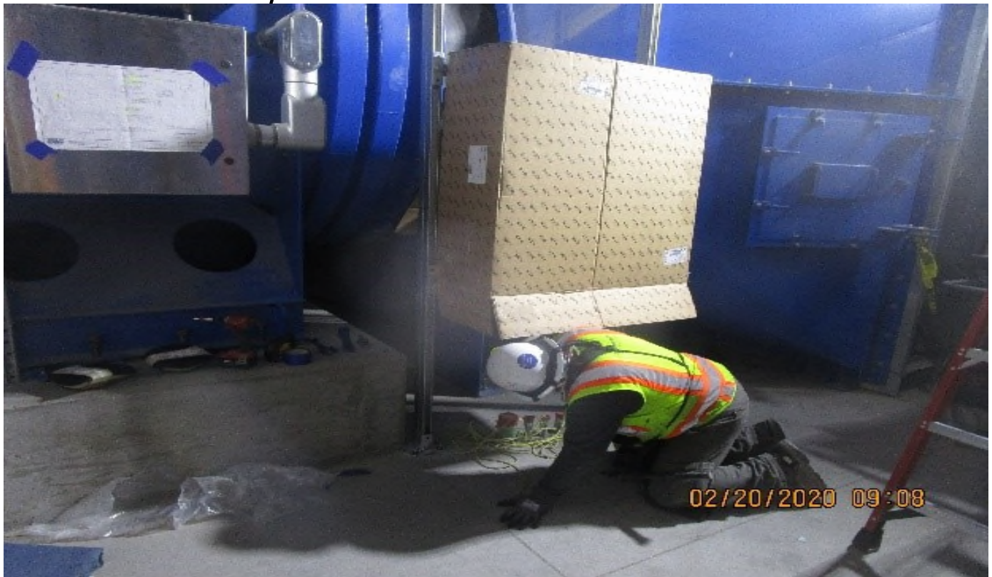
MLK STATION – Emergency Fan room (S) EVF-7-321 Continued at pull box 2 of 2 rough in supports per non approved plan.
