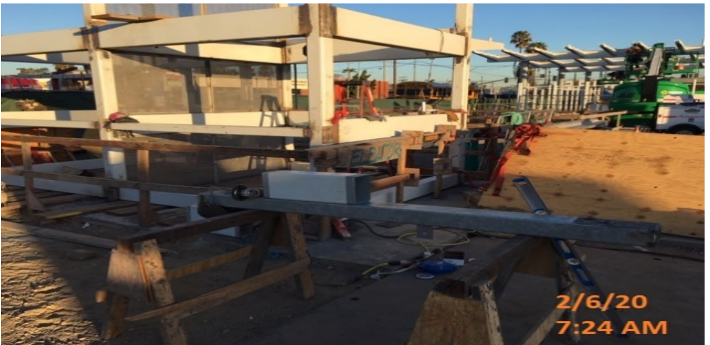
EXPO STATION – Installing and welding HSS members of door frame of Elevator structures 1&2 at the plaza level.
