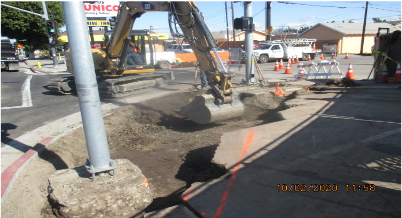
UG3 – Excavating and removing temporary AC for new installation and concrete placement of sidewalk and ADA ramp on the southeast corner of 67th St and Crenshaw Blvd. 2/10/20
