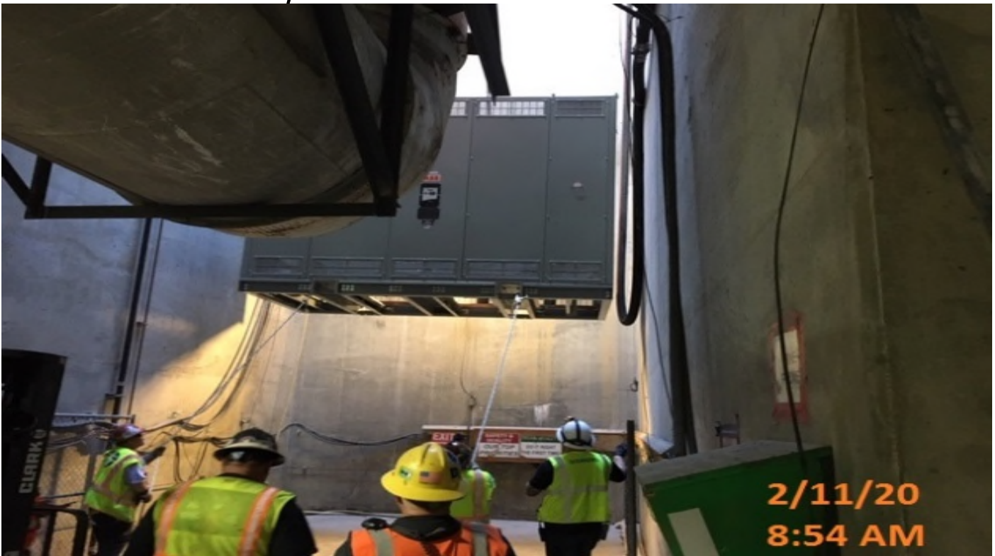
EXPO STATION – Placing transformer on top of dielectric pad in the TPSS Room T – 115
