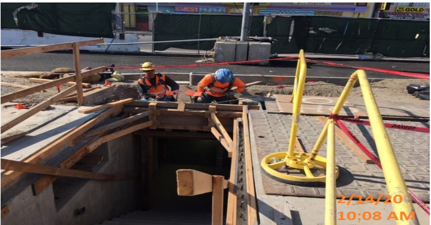
LEIMERT PARK STATION – Began imbed and hydrophilic water stop installation for Emergency Exit Hatches 1&2 at the plaza level.
