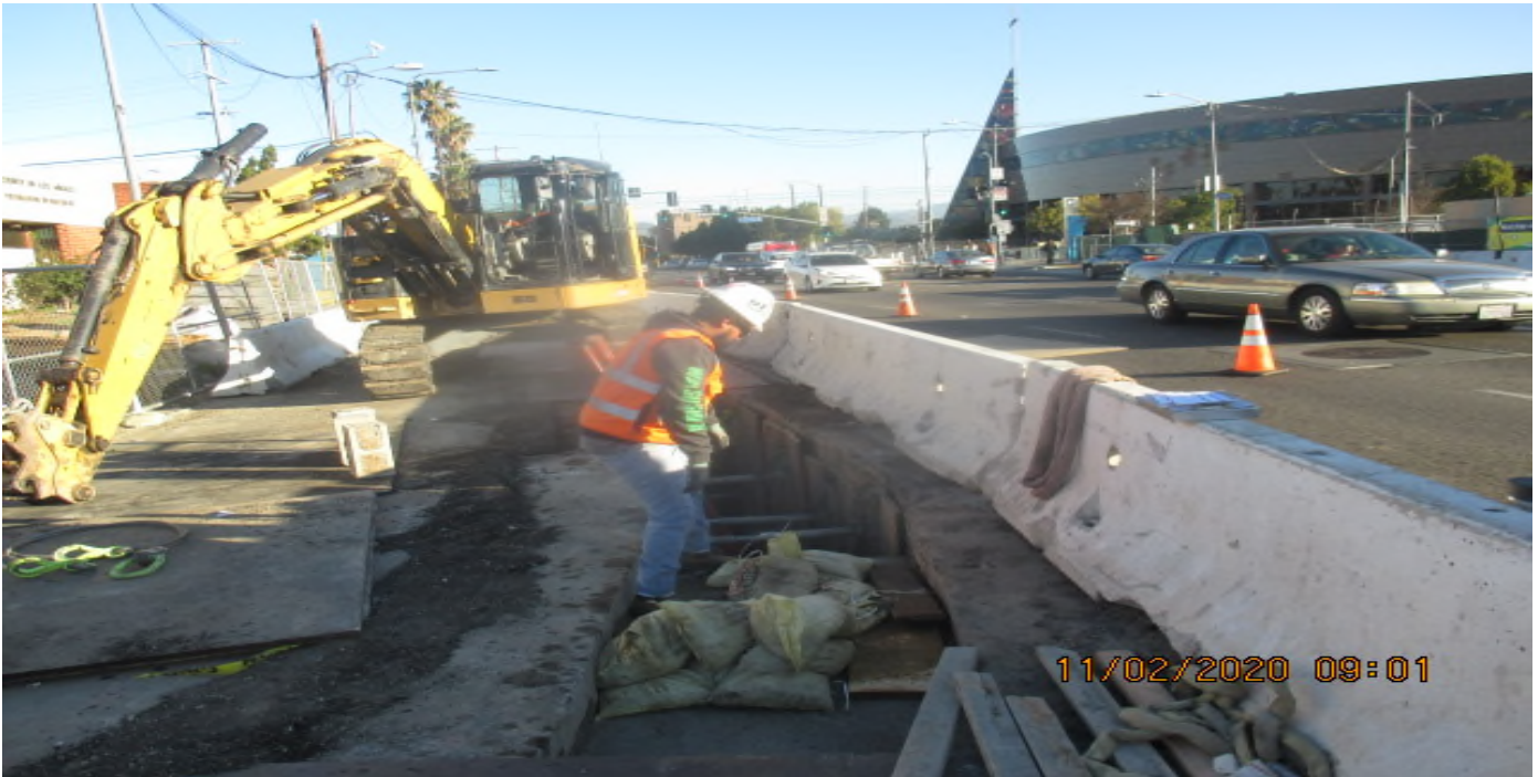
EXPO STATION – Continued installing sections of the 24” RCP for Line W – storm drain on the northbound side of Rodeo Blvd and Crenshaw Blvd. 2/11/20
