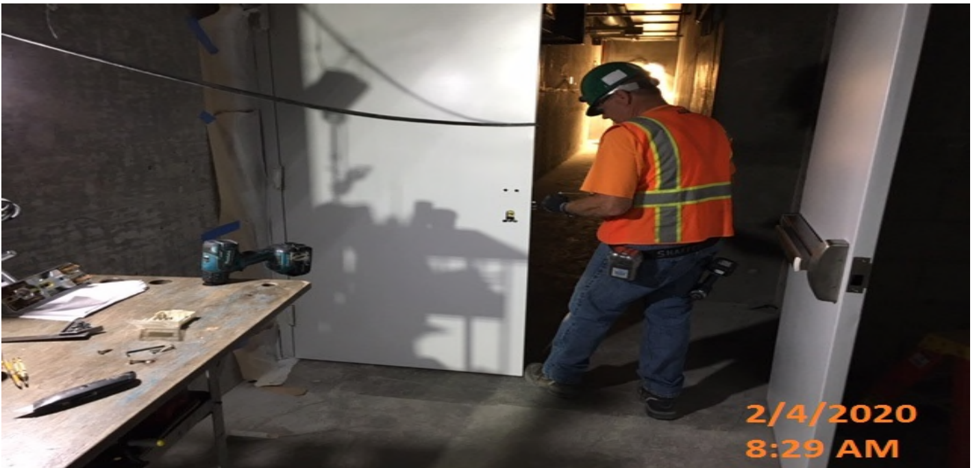
EXPO STATION – Reinstalling hardware on all completed painted doors at the concourse level.
