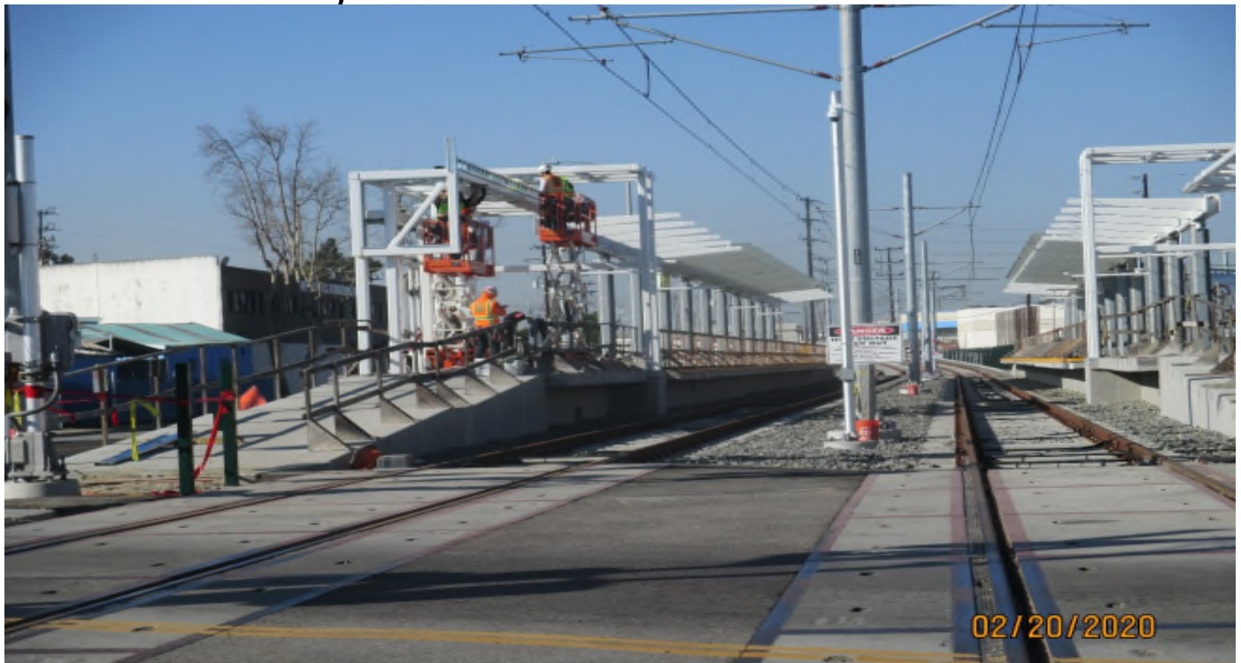
HINDRY AVE- Metal stud installation on the NB Hindry Station platform TVM.
