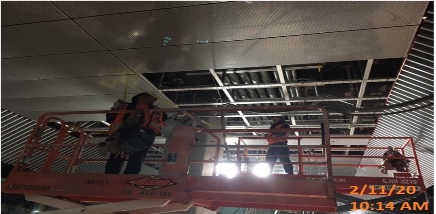
LEIMERT PARK STATION – Continue installing metal ceiling panels above the platform level.
