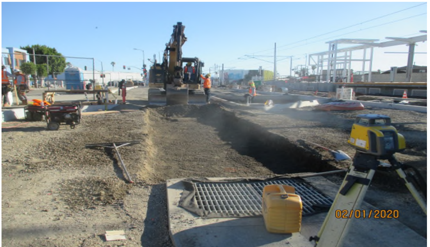
WEST STATION- Cross gutter grading at the West Station park and ride.
