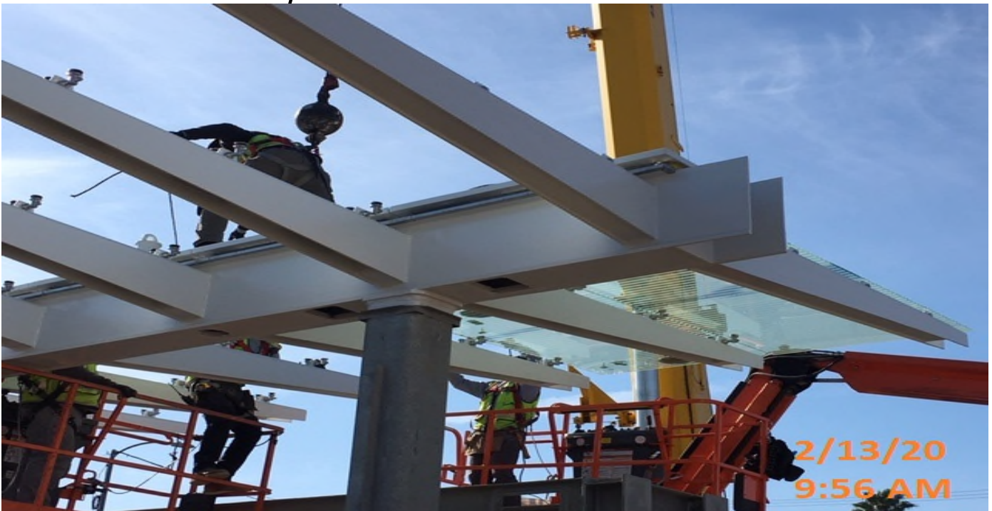
LEIMERT PARK STATION – Began glass panel installation for the main entrance canopy structure at the plaza level.
