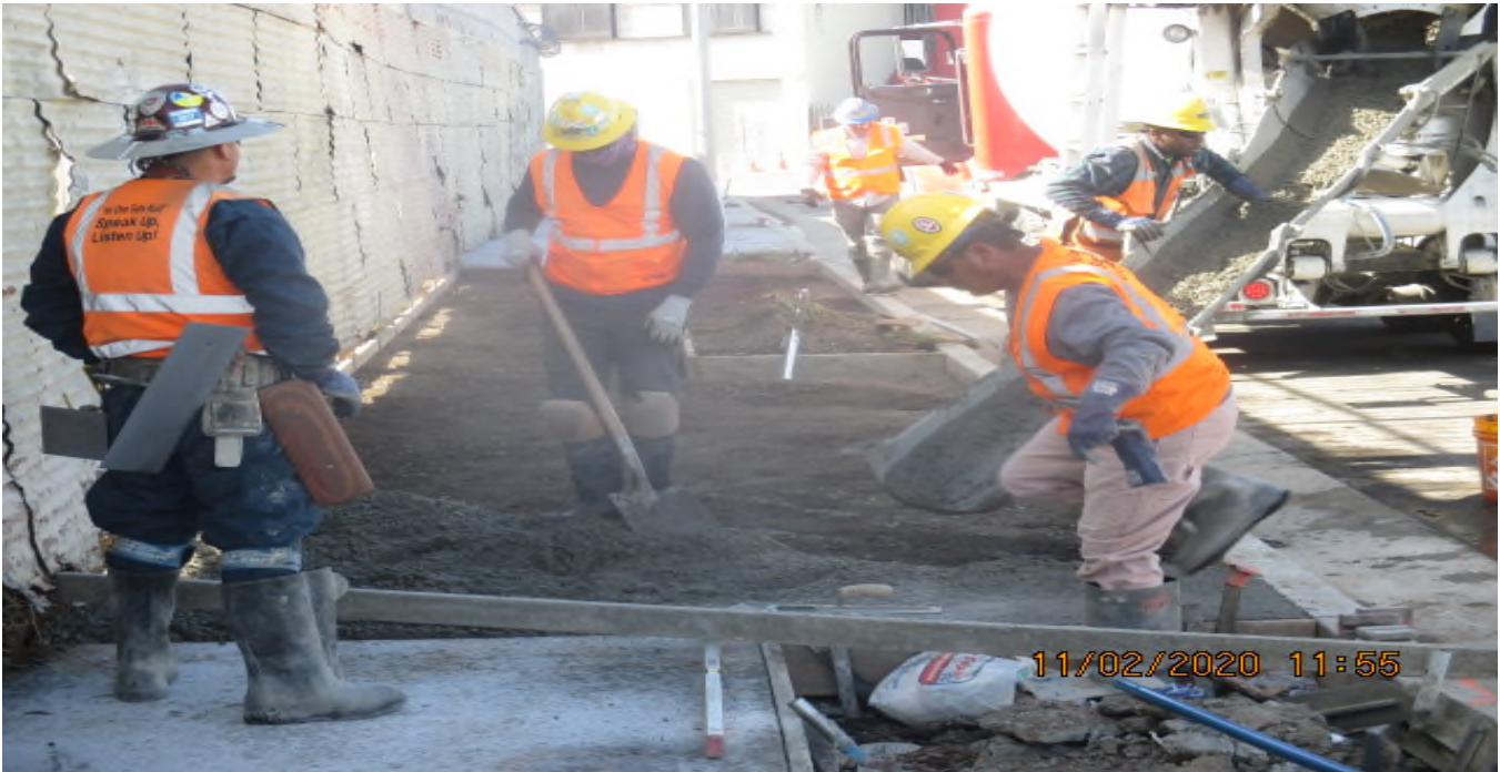
UG3 – Began concrete placement on both west and eastbound “New Road” sidewalks. 2/11/20
