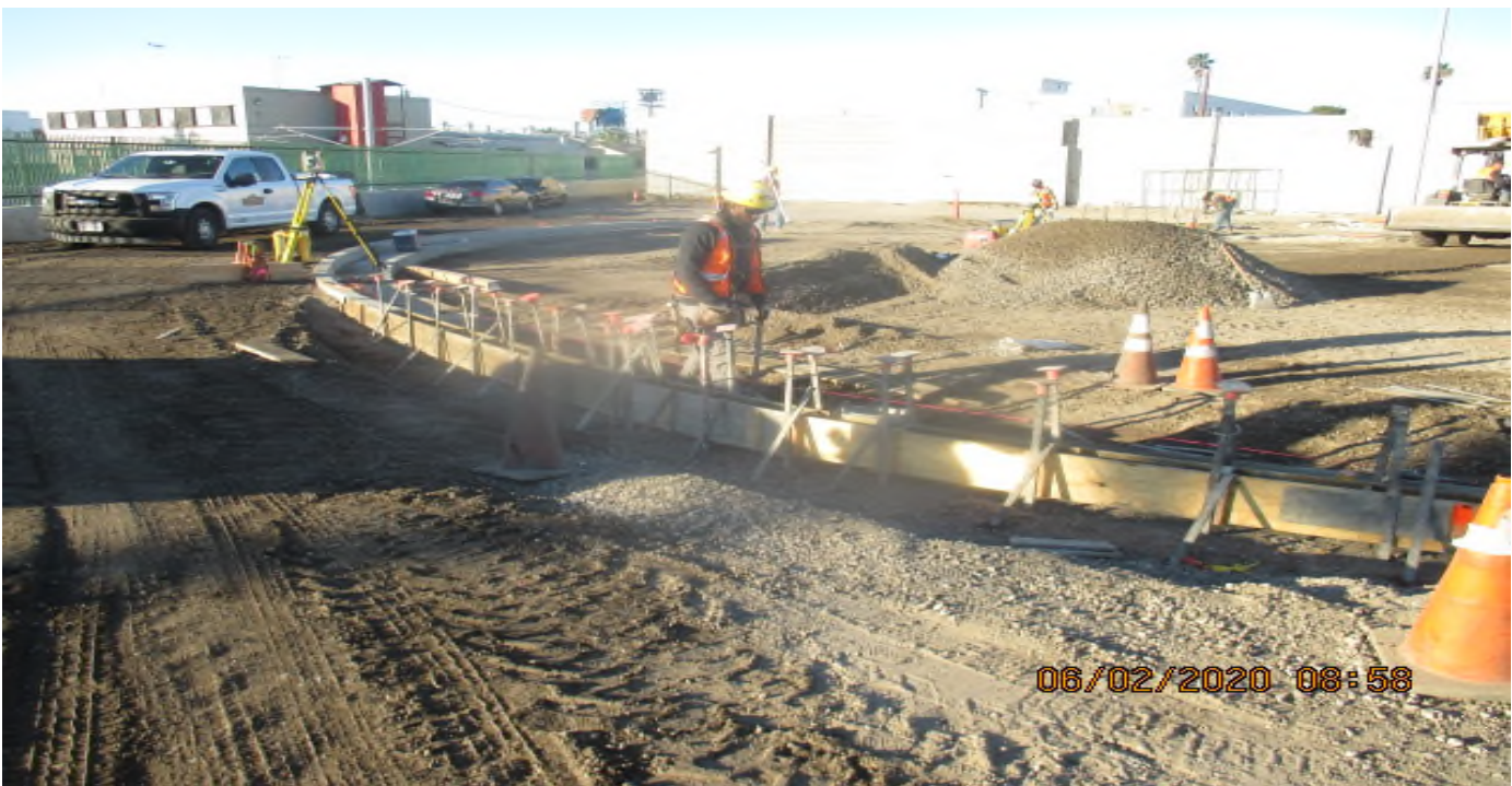
UG3 – Continued excavation/compaction of the new Cul-de-sac in preparation for curb/gutter installation and concrete placement at North Victoria Ave. 2/6/20
