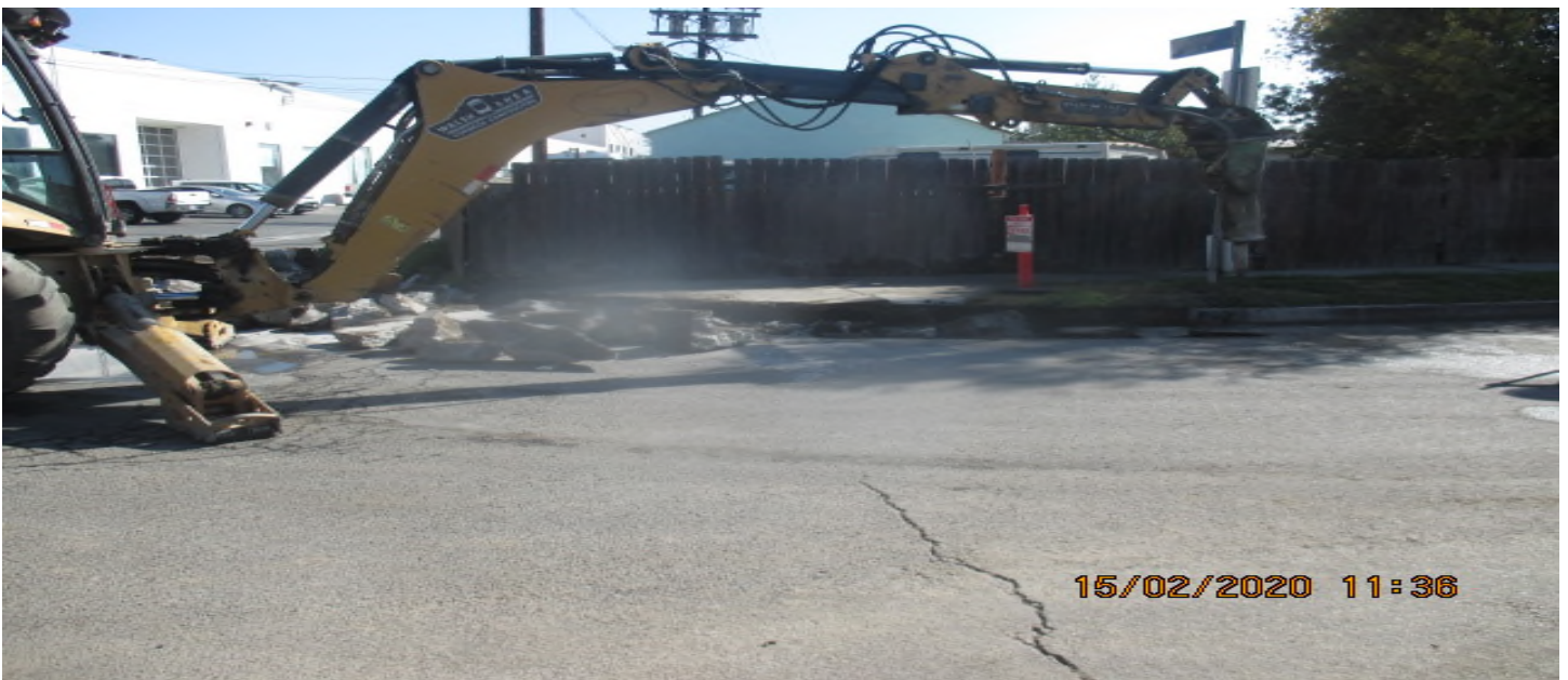
EXPO STATION – Continued demolishing and excavating curb/gutter for the new Cul-de-sac construction on Bronson St. east of the plaza. 2/16/20
