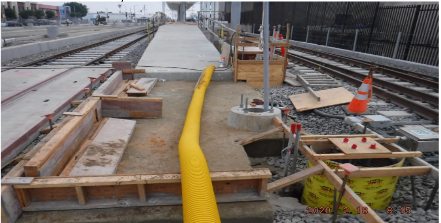
WEST STATION- STA262+75_ looking North_ Landing pad & foundation vacuum excavation status_PUNCH LIST_West
