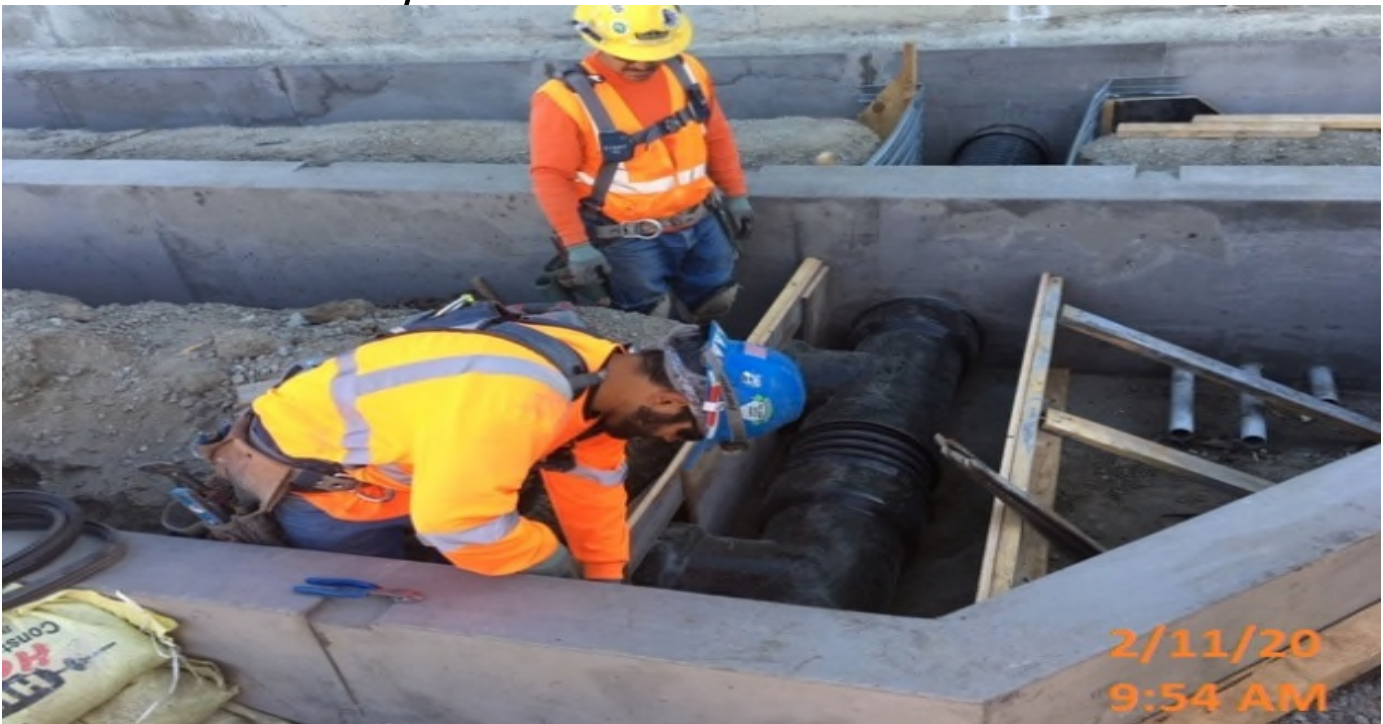
LEIMERT PARK STATION – Building formwork for slurry encasement of 12” HDPE drainage pipe at the plaza level.
