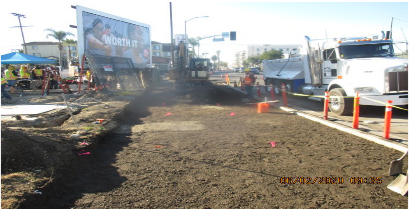
Park Mesa – Continued excavating for new concrete sidewalk installation on the northeast corner of 60th St & Crenshaw Blvd. 2/6/20
