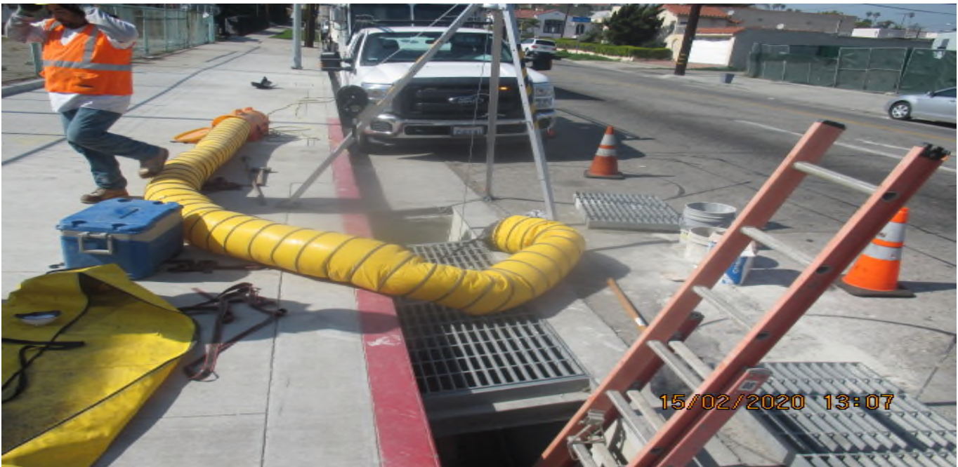
Park Mesa – Sack and patch of Catch Basin #36 on the southwest corner of 48th St and Crenshaw Blvd. 2/15/20
