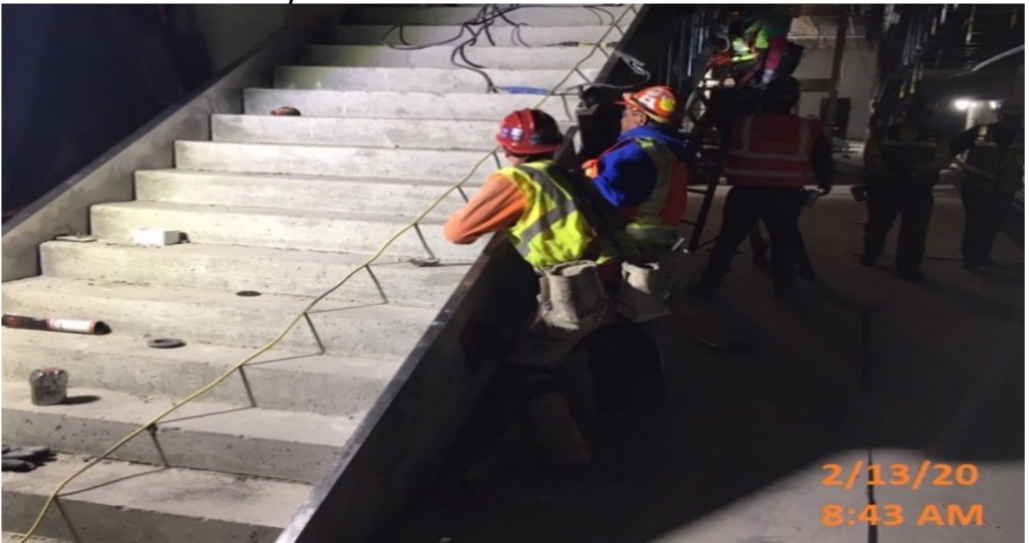
EXPO STATION – Continued edge plate installation for staircase 3 at the platform level.
