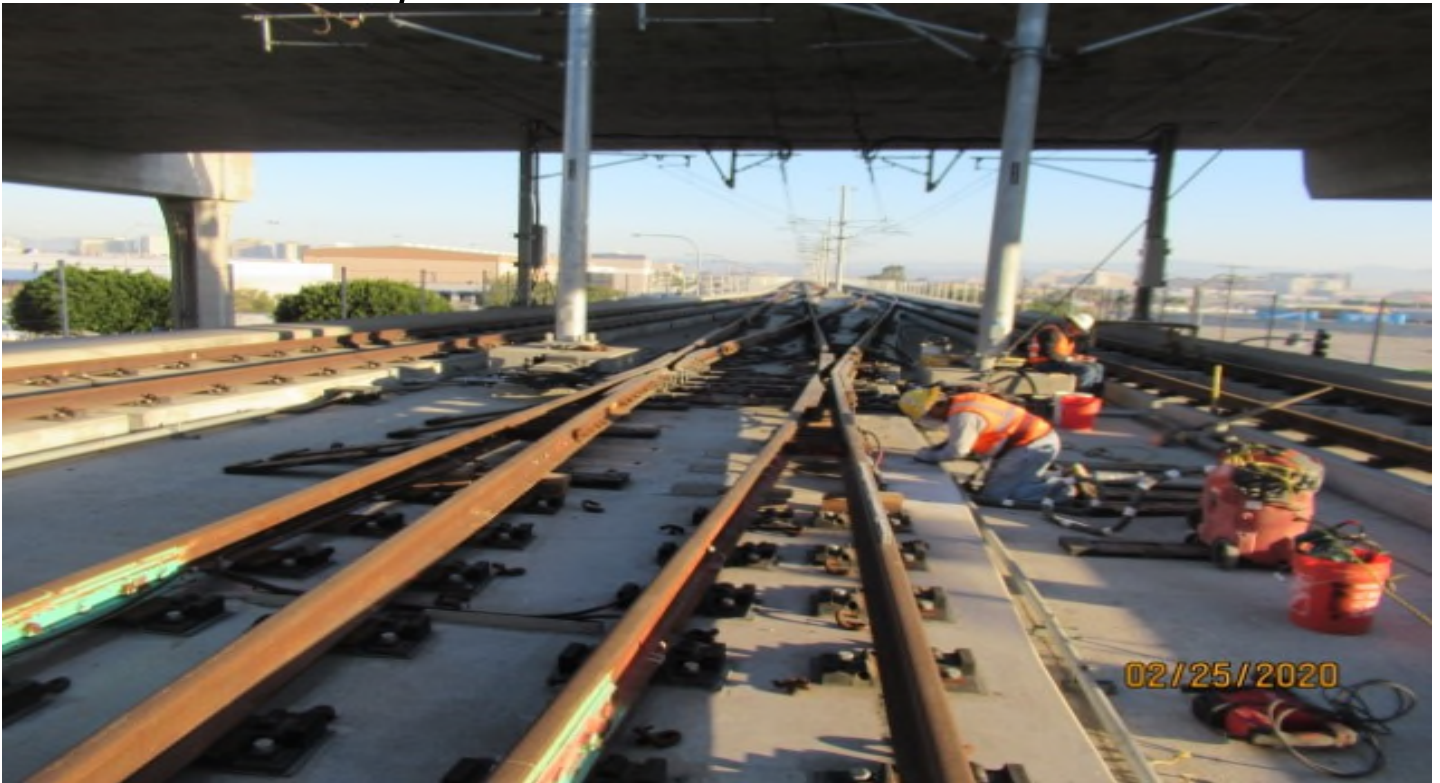
GREENLINE UNDERPASS - WSCC working on evening out concrete slab for MPF southeast portion GL Wye STA 13+90
