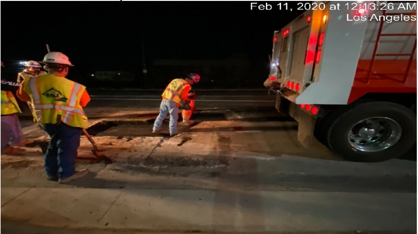
Park Mesa – Paving road on top of LADWP main line tie-in at the intersection of 60th St & Crenshaw Blvd.
