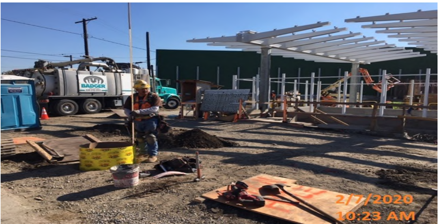
LEIMERT PARK STATION – Setting sonotubes in preparation of concrete placement for the footing of the luminaire light posts at the plaza level.
