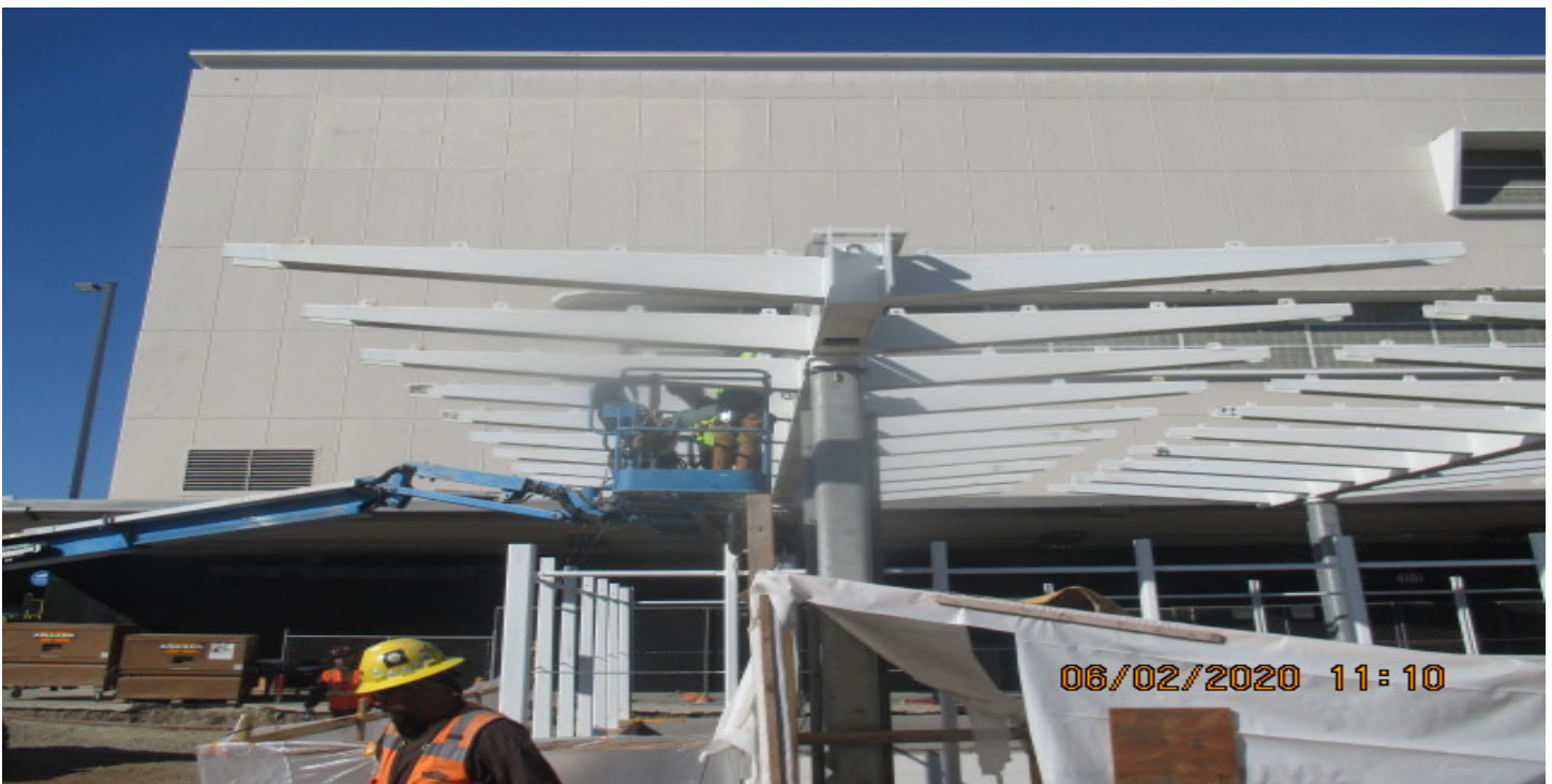
MLK STATION – Continued catwalk and gutter installation on top of the main entrance canopy structure at the plaza level. 2/6/20
