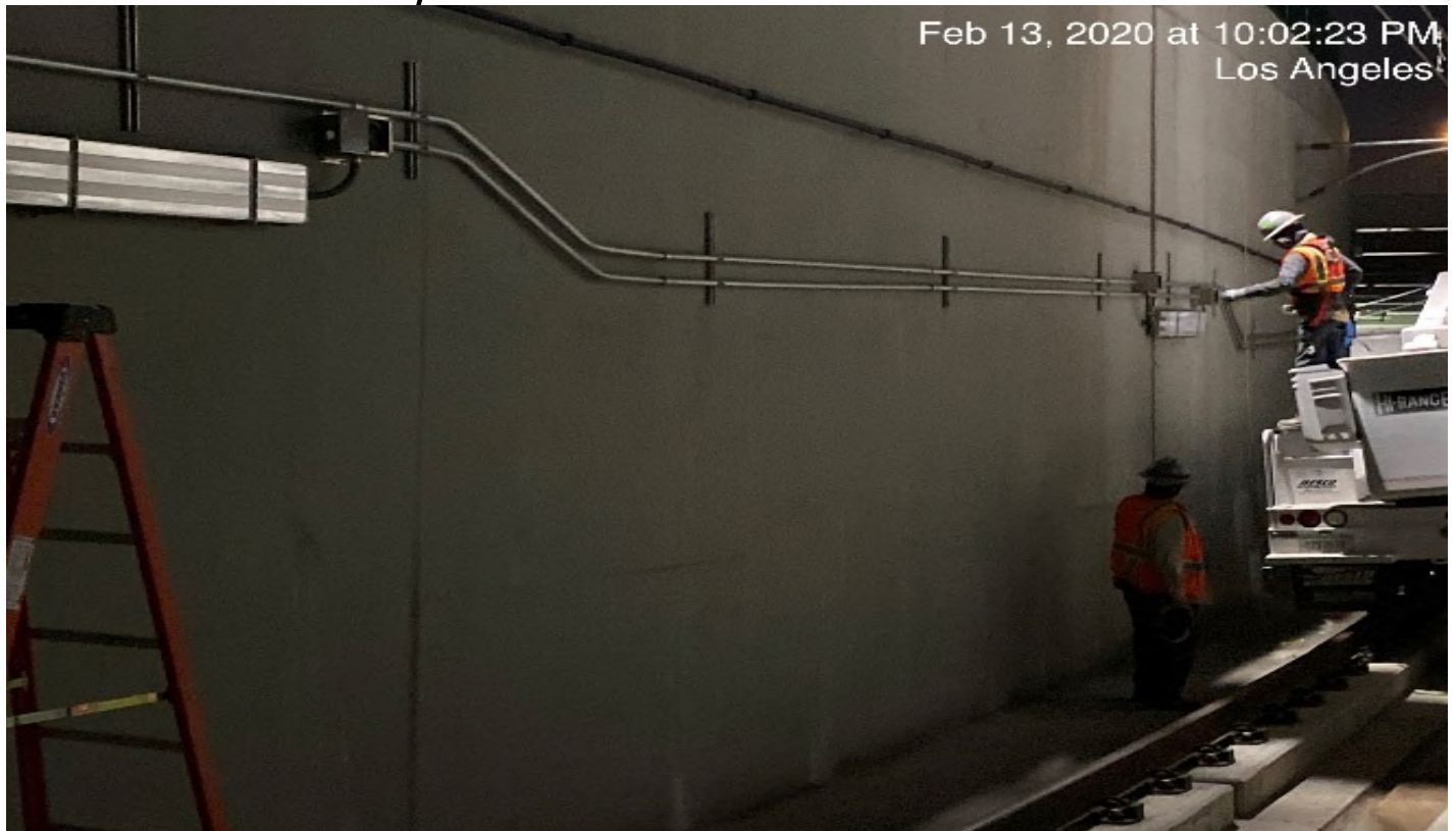
UG3 – Continue pulling wire for the emergency lighting at the south end portal entrance.
