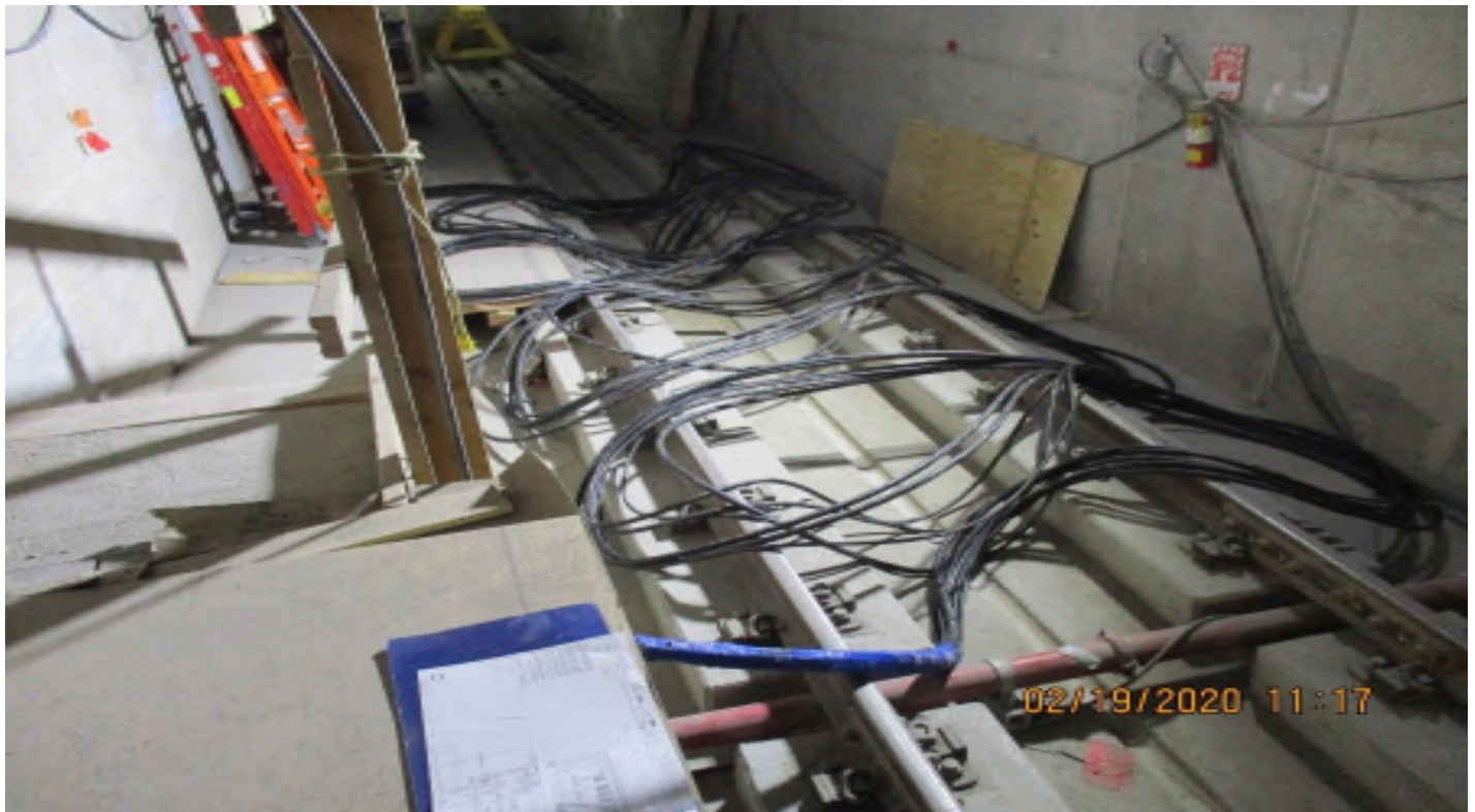
EXPO STATION- LKC Personnel Pulled Cable Adjacent to the South Cable Room, Looking West.
