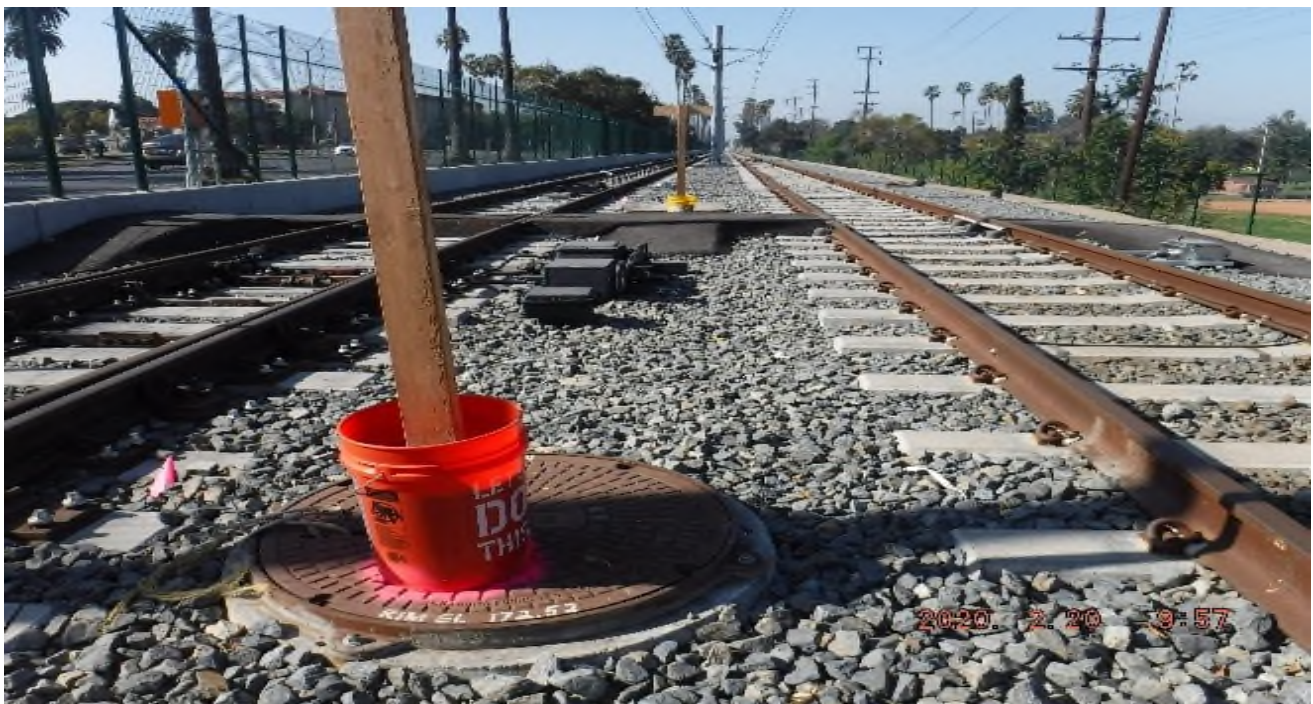
HIGH STREET- STA 244+74 NB looking south – MH#68 rim elevation vs. TOT; no track work (Centinela – High)
