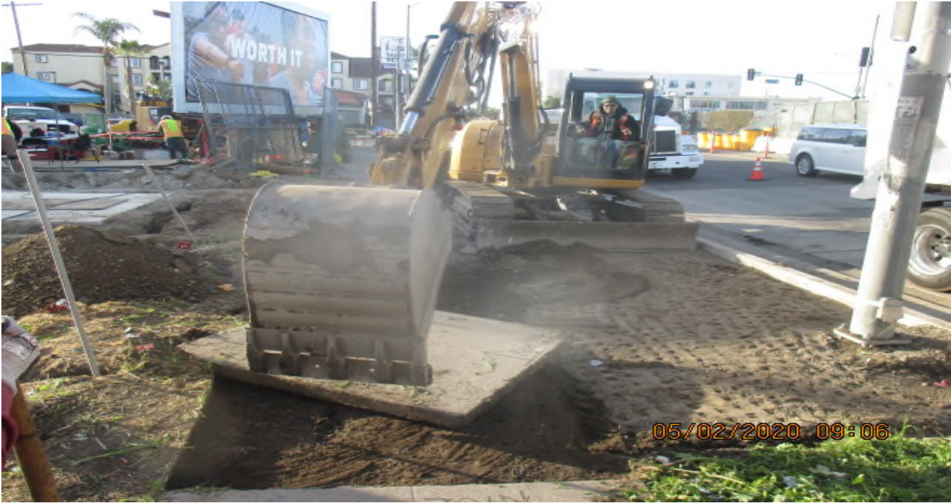
Park Mesa – Excavating for new concrete sidewalk installation on the northeast corner of 60th St & Crenshaw Blvd. 2/5/20
