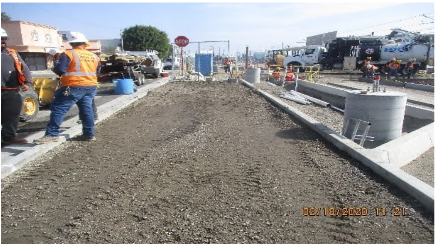
WEST STATION- WSCC Making fine grade for asphalt and SWK at West Sta park and ride.
