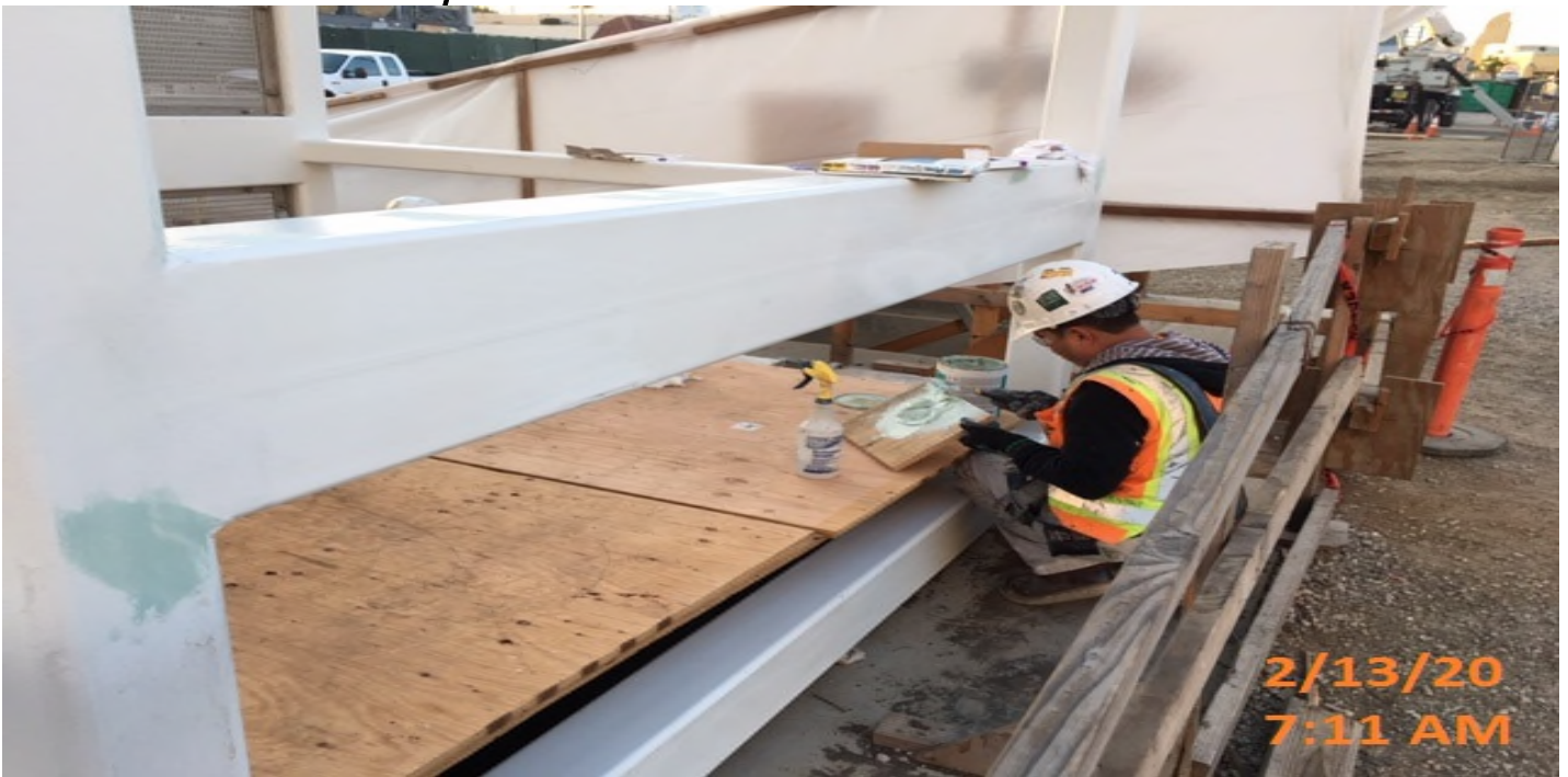
MLK STATION – Preparing for primer application for Elevator structures 1&2 at the plaza level.
