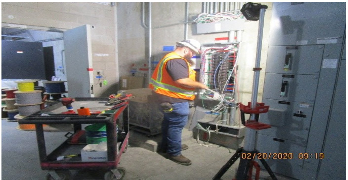
MLK STATION – Aux Power (N) C132, Distribution panel VP1A-N Continued dressing & terminating FSD power.
