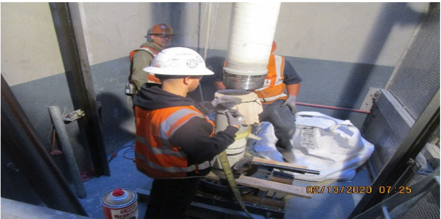
LEIMERT PARK STATION – Continued jack installation inside Elevator hoist way/pit 1 at the concourse level.
