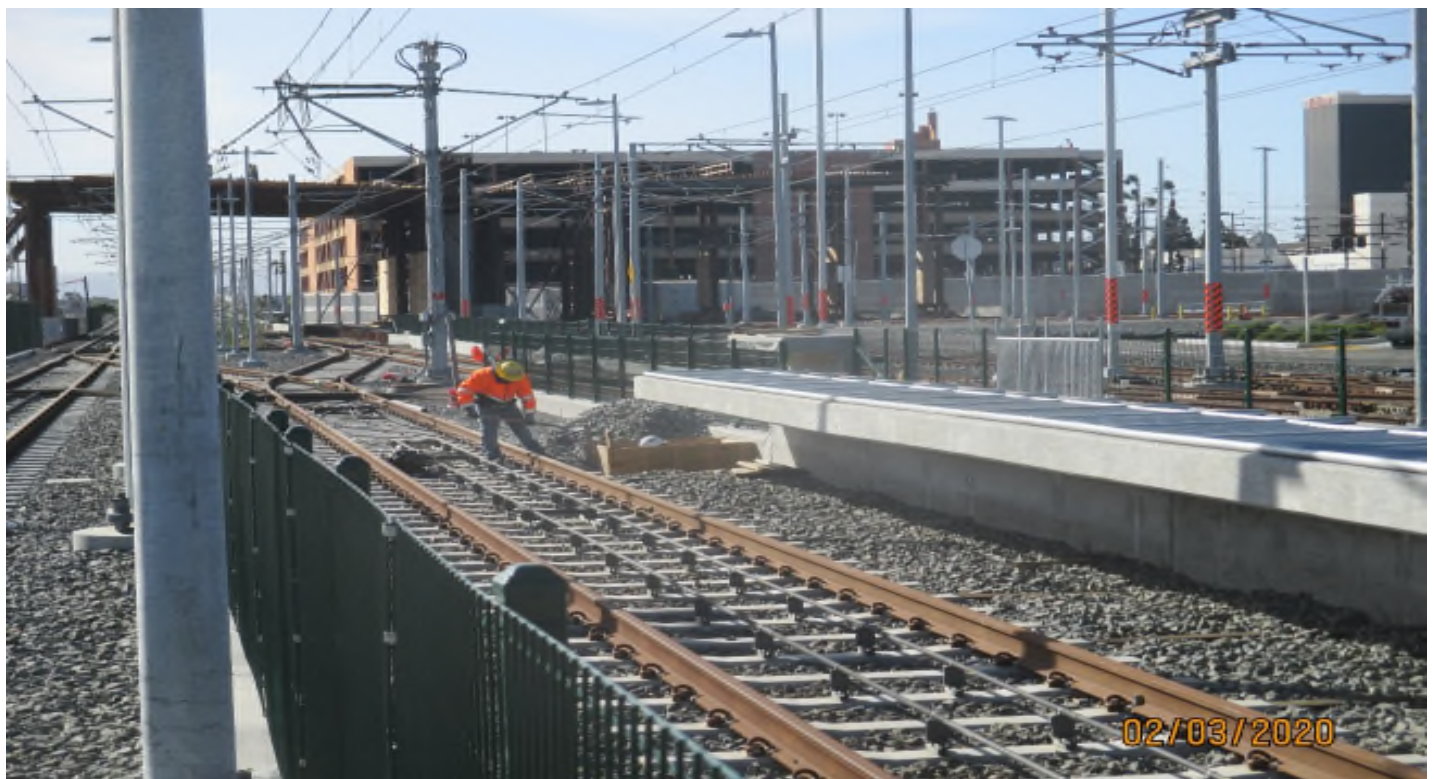
96 th STREET- Excavating the ballast the set forms for the operators platform stairs.
