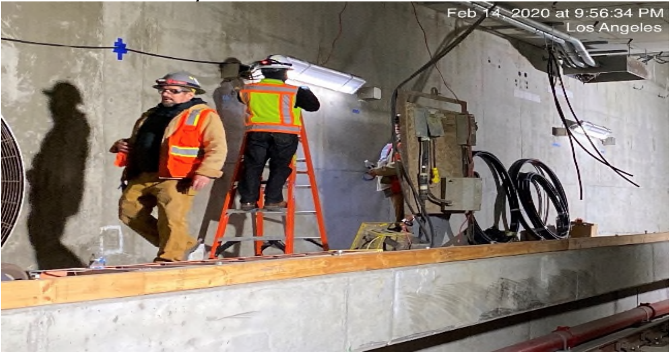
UG-4- Continue pulling wire for the emergency lighting at the south end portal entrance.
