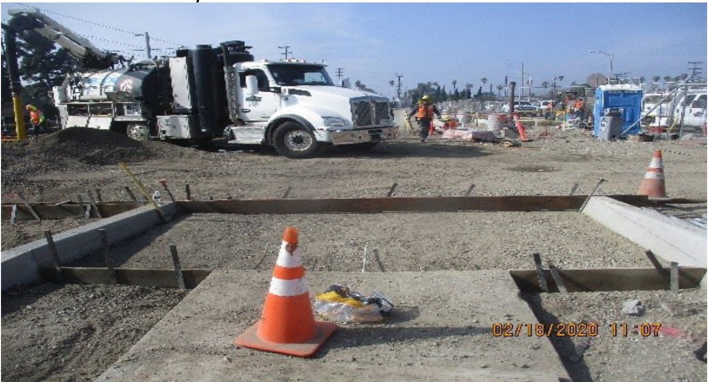
WEST STATION- WSCC Placing conc curbs and gutter at West Sta Park and Ride.
