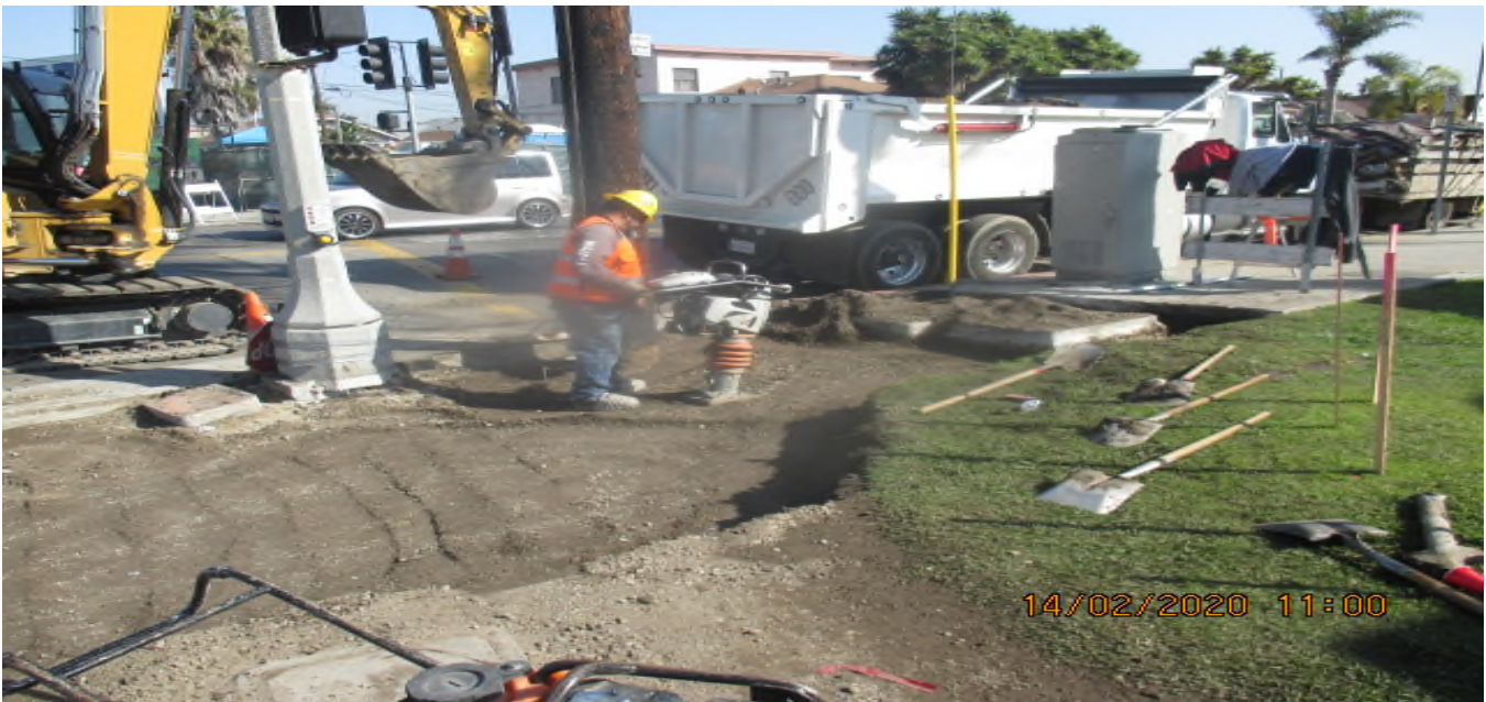
Park Mesa – Continued excavating for new concrete sidewalk installation on the northeast corner of 60th St & Crenshaw Blvd. 2/6/20
