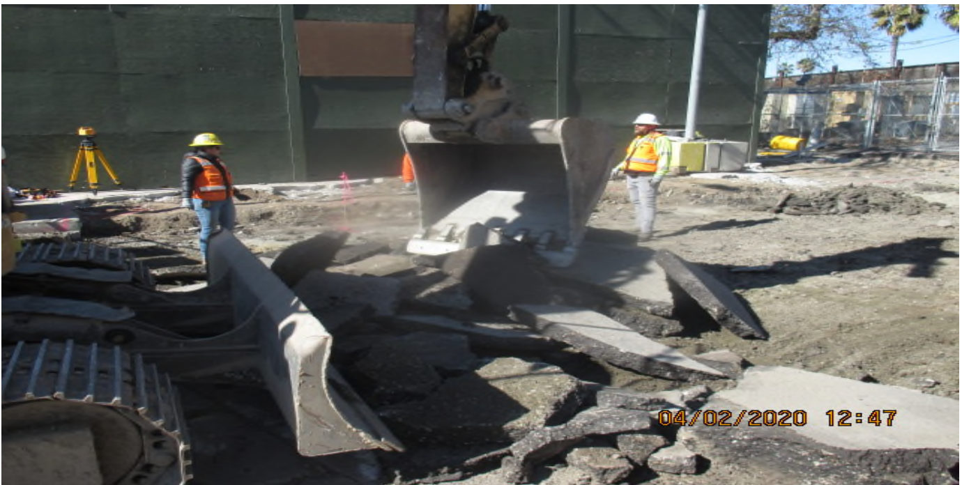
EXPO STATION – Demolishing and excavating for the new Cul-de-sac construction on Bronson St. east of the plaza. 2/4/20
