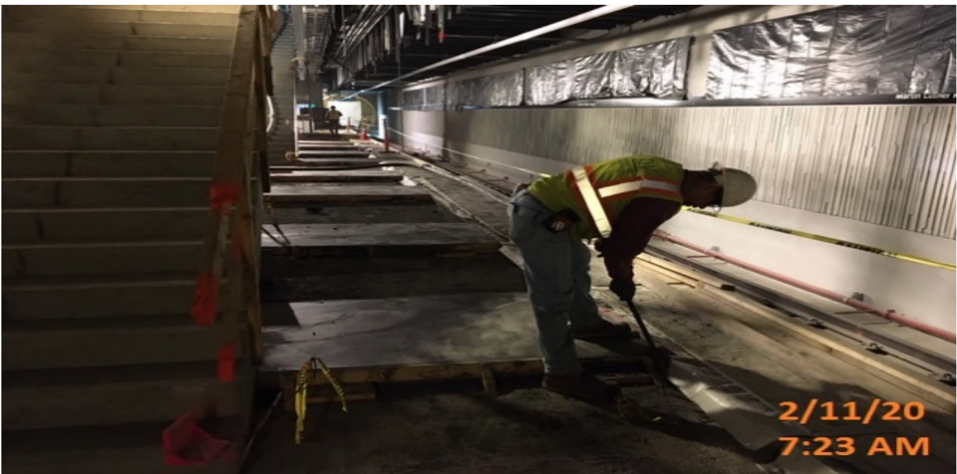
MLK STATION – Removing formwork and setting up for 2nd phase of concrete placement of the architectural topping slab at the platform level.
