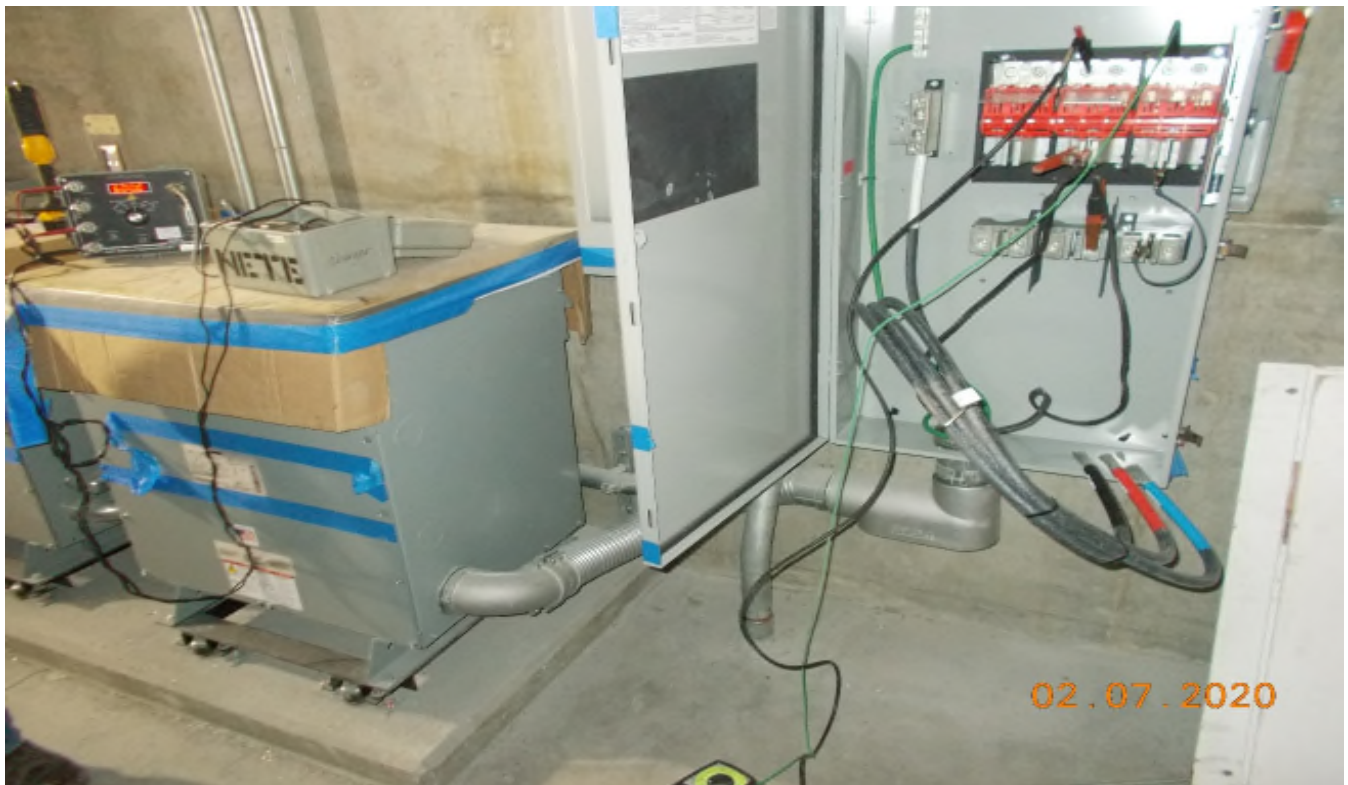
VERNON STA – NETE was testing the disconnect switches in the TCC room.
