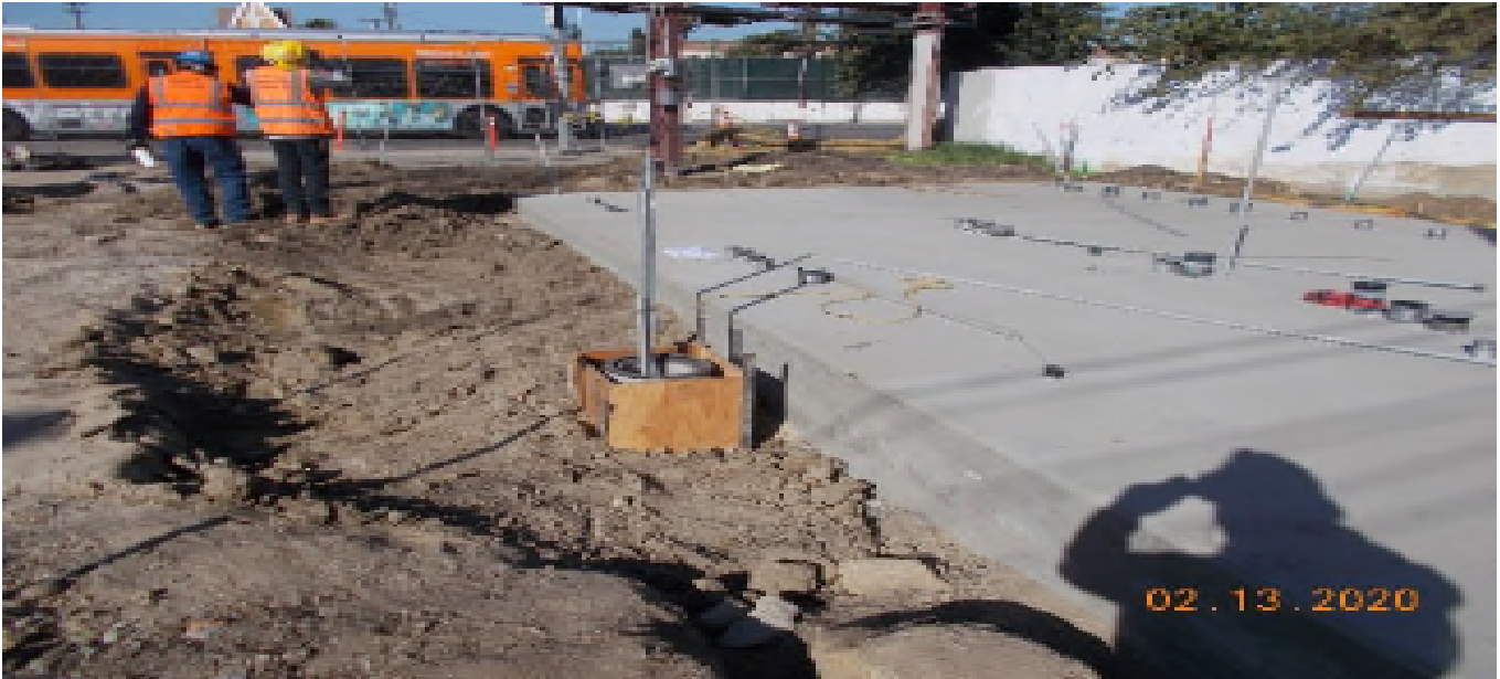
Park Mesa – Grading in preparation for the placement of the auxiliary power bungalow and generators on top of equipment pads at 60th St & Crenshaw Blvd.
