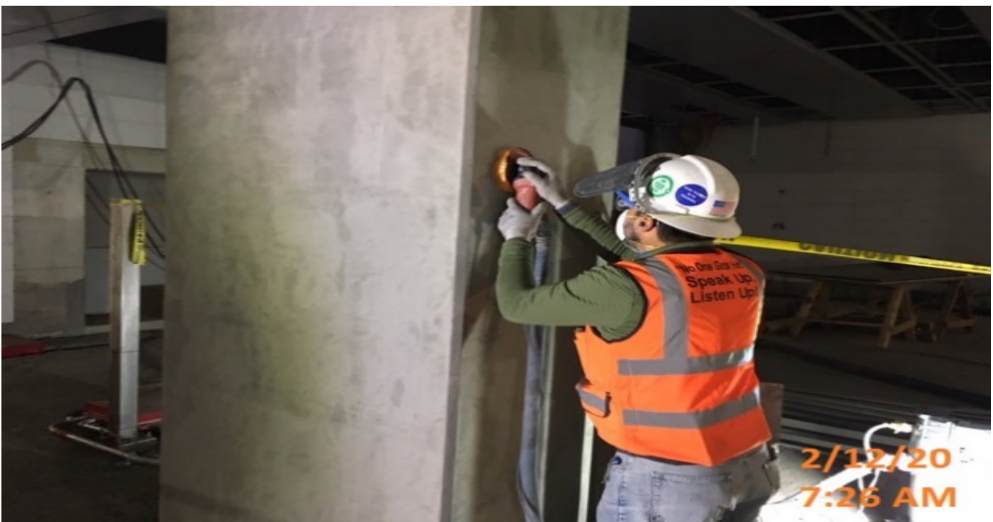
MLK STATION – Grinding and smoothing columns in the Free Area of the concourse level.
