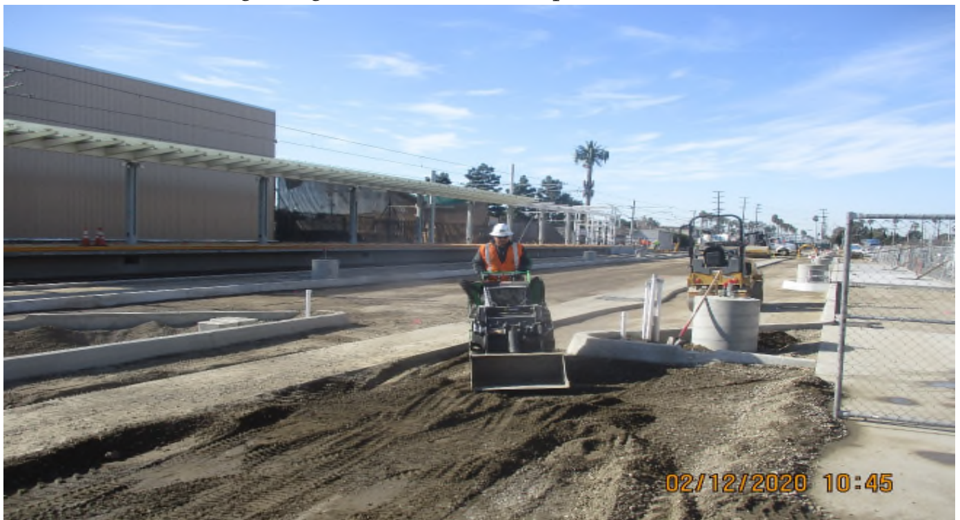
WEST STATION- WSCC Making fine grade for asphalt at West Sta parking lot.
