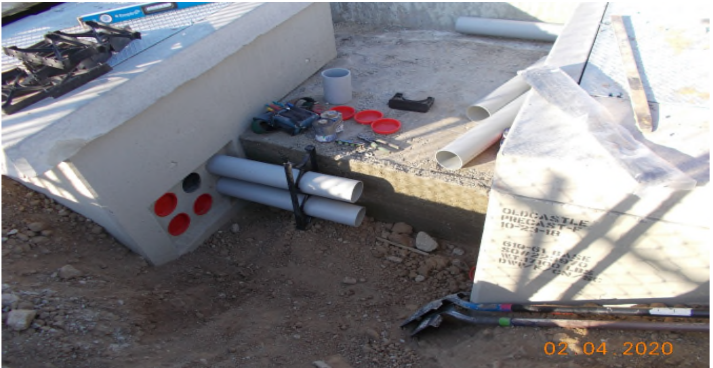
104th St. Substation - Dyna Electric was installing two 5-inch conduits between the DWP precast boxes
