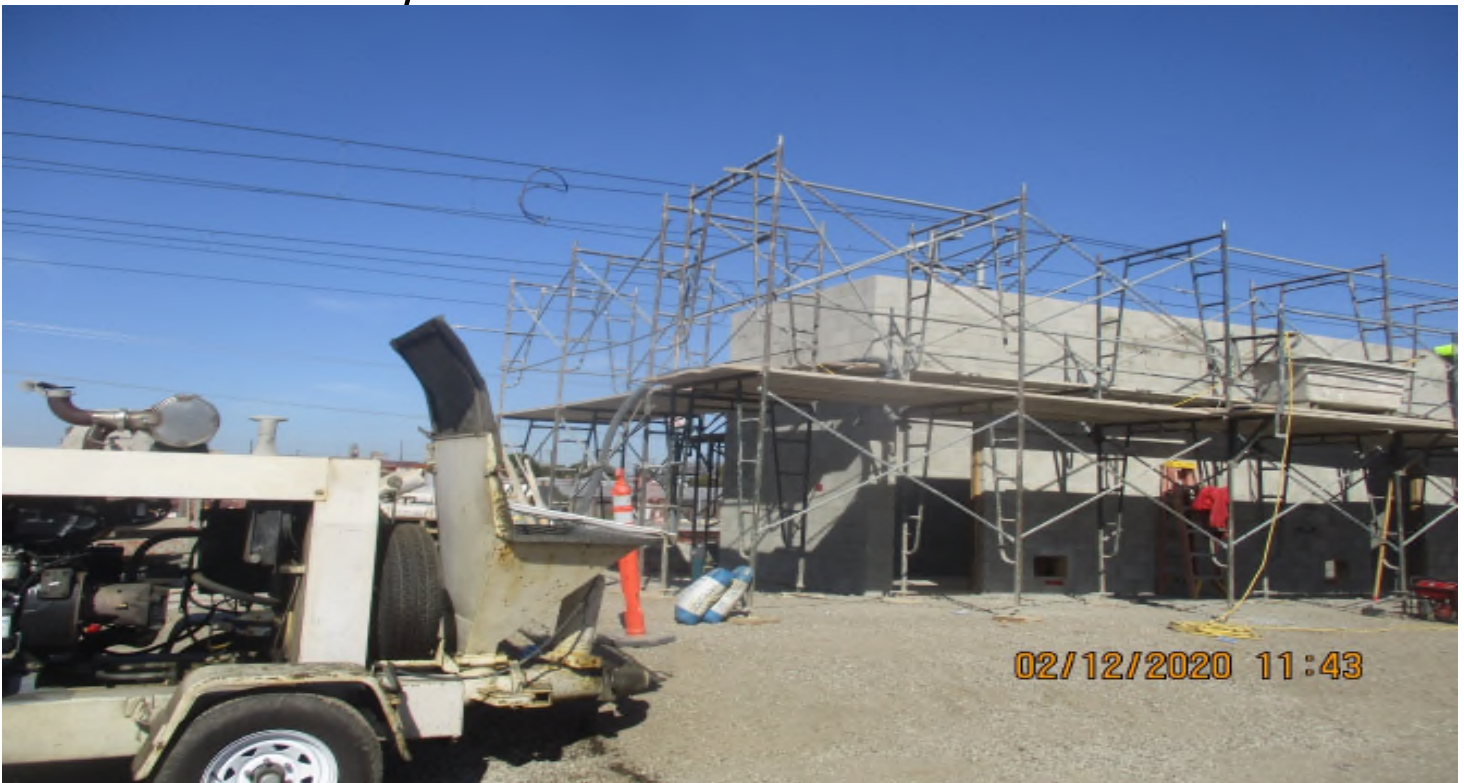
LA BREA – Masonry Concepts Placing grout in block walls at La Brea bathrooms.
