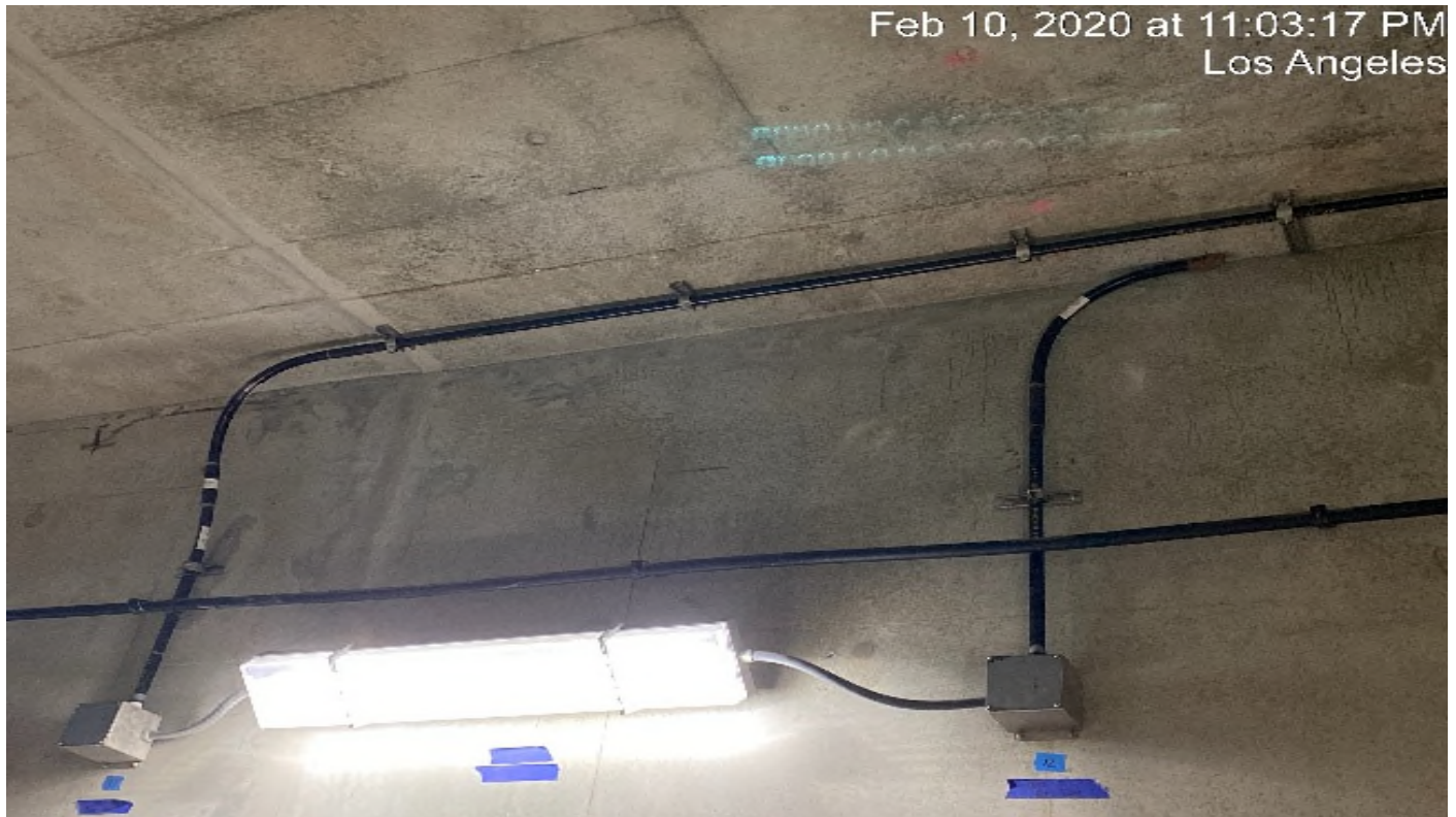
UG3 – Placing phenolic conduit for the emergency lighting at the sump pit area.
