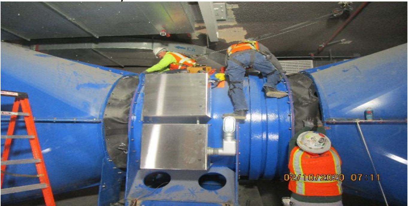
LEIMERT PARK STATION – Continued installing silicone gaskets and roughing in flex connectors to EVF-6-102 in the North Fan Room C – 126 Fan Rooms of the concourse level.
