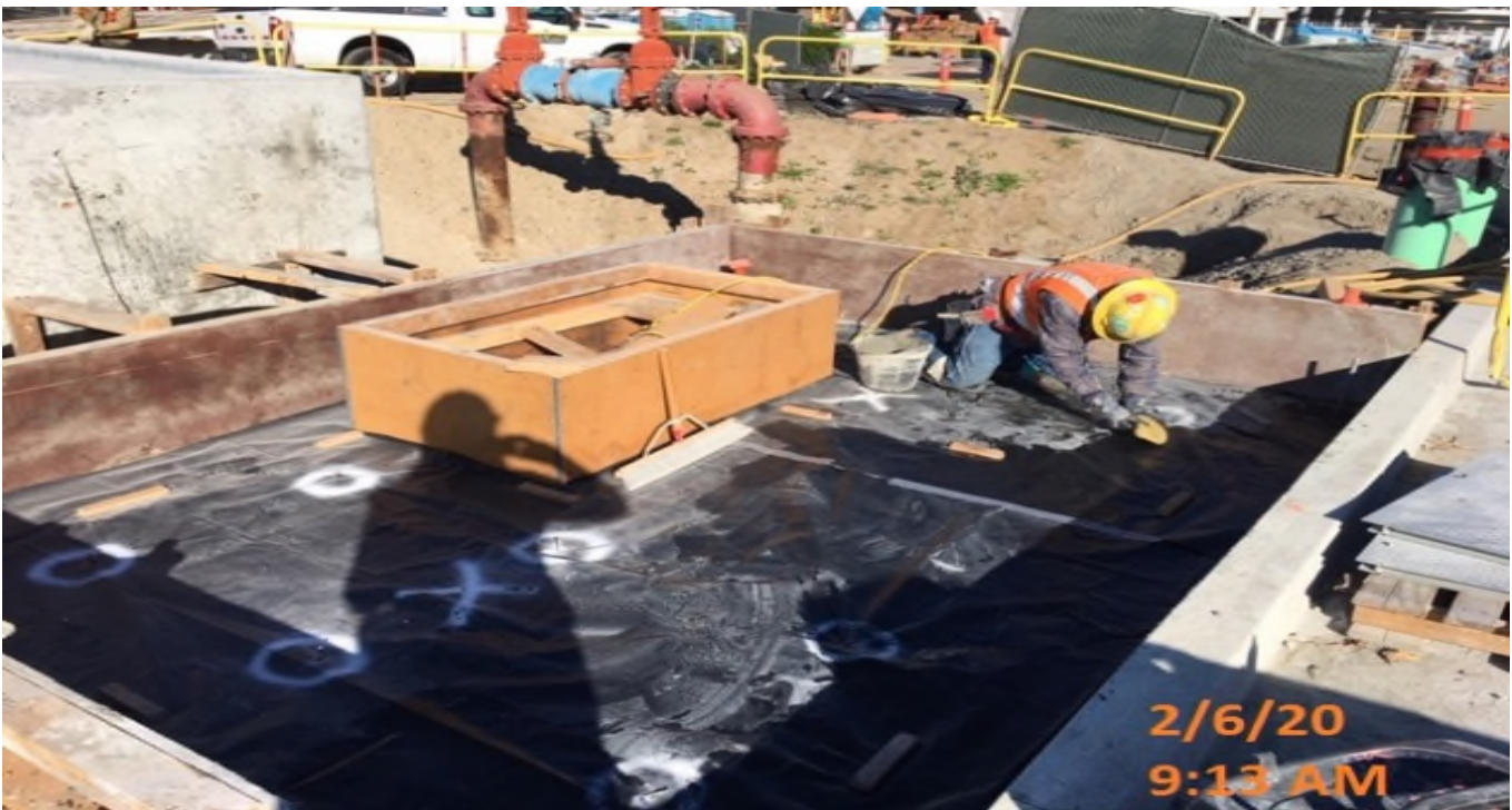
MLK STATION – Prepping valve pit access hatch formwork for concrete placement at the plaza level.
