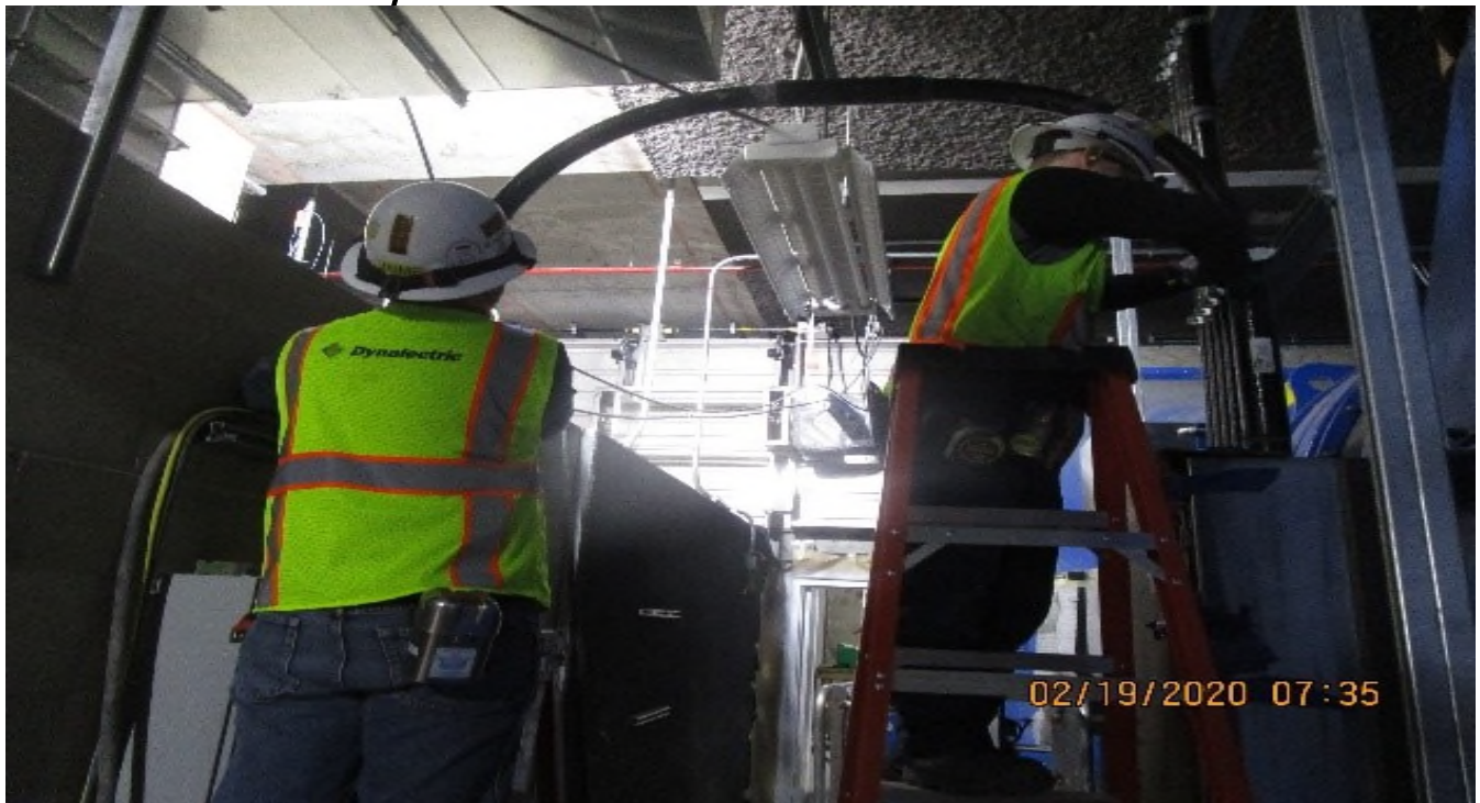
VERNON STA – Emergency Fan room (S) C102, EVF-6-101, continued (3) 2" FRP from PB 1 of 2 to EVF control panel
