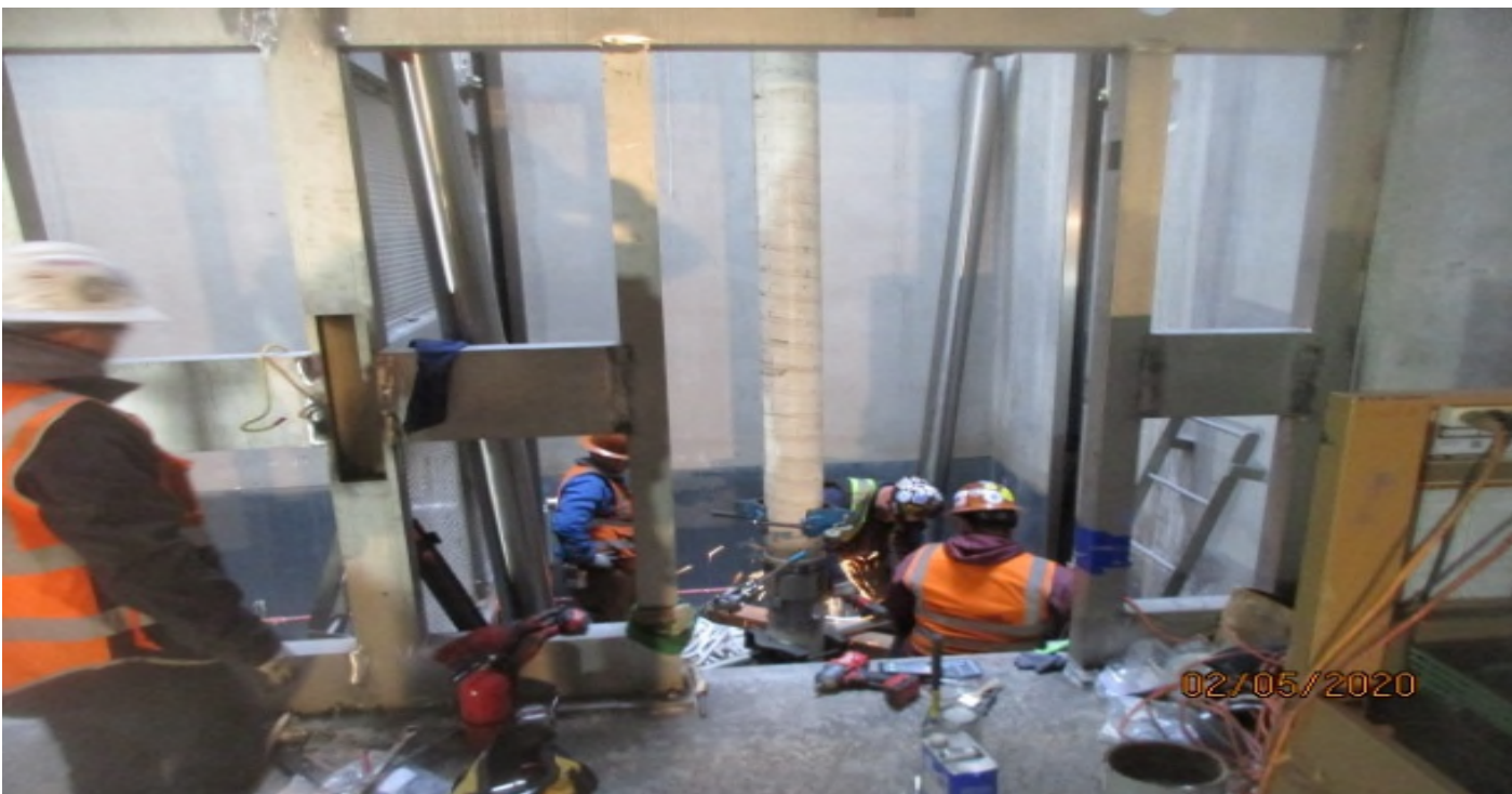
MLK STATION – Continued jack installation inside Elevator hoist way/pit 1 at the concourse level.
