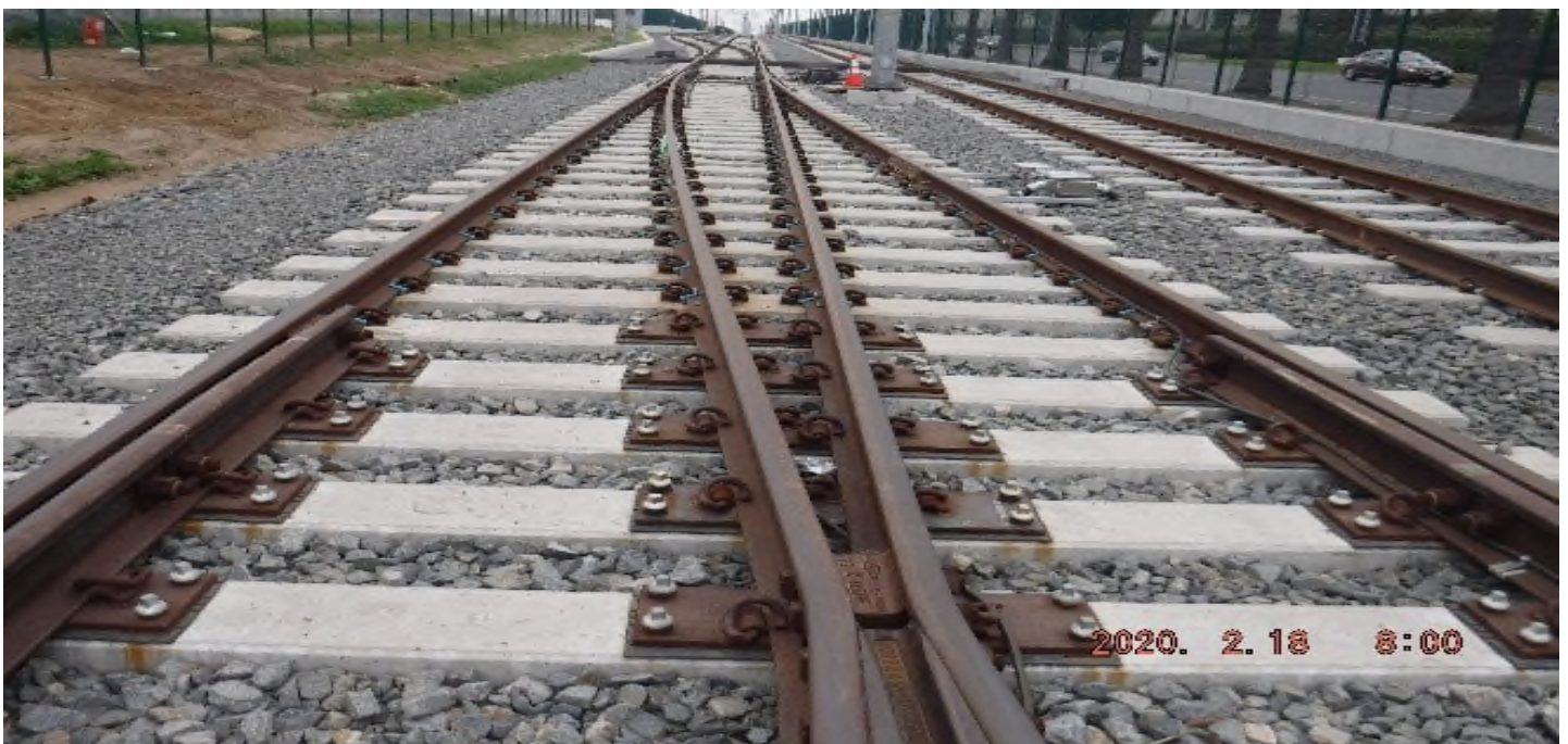
HIGH STREET- STA 245+92 SB looking north – frog of 10Q2LHXO new spike screws (Prairie- High) PUNCH LIST
