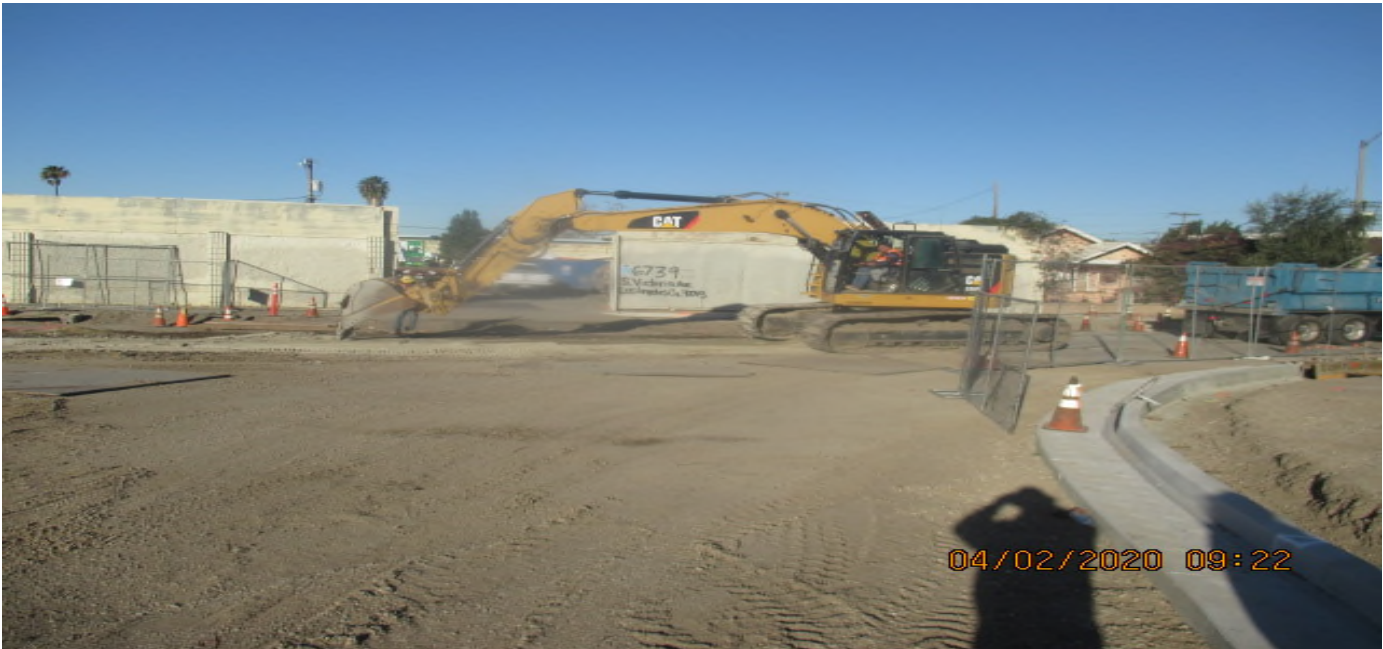
UG3 – Continued excavation/compaction of the new Cul-de-sac in preparation for curb/gutter installation and concrete placement at North Victoria Ave. 2/4/20
