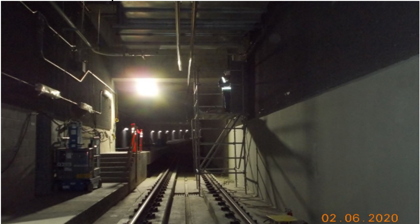
VERNON STA – Faith Electric was racking and securing a high voltage wall box on track #3 near the platform
