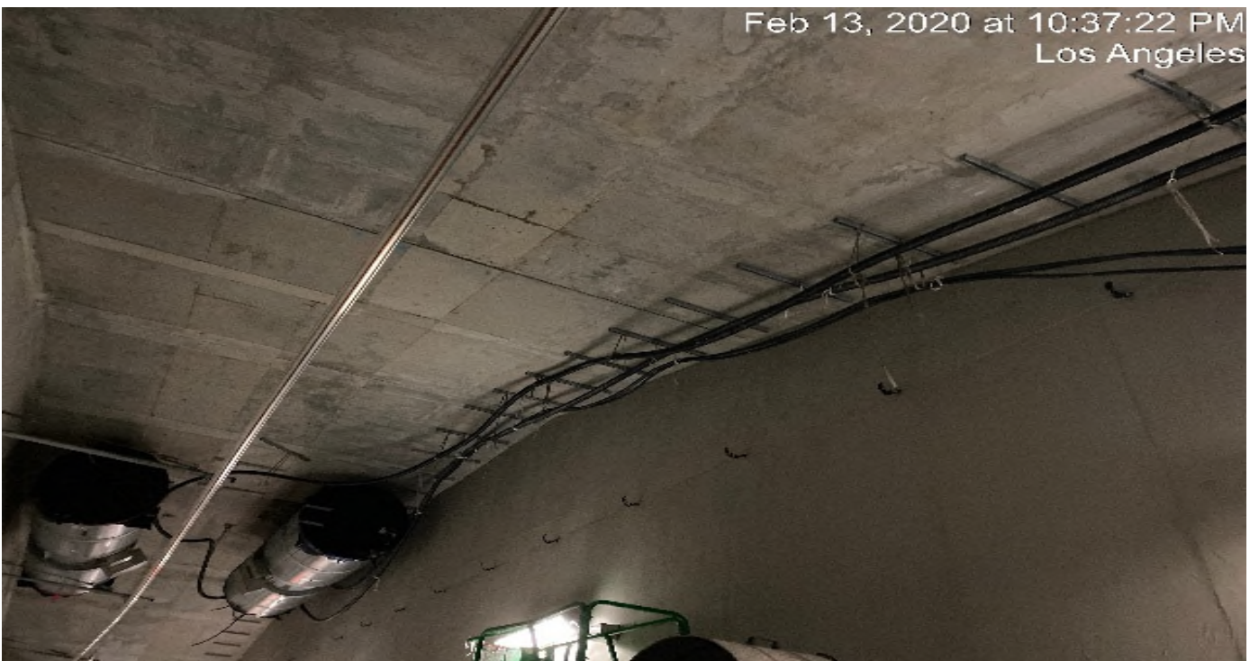
UG-4- Continue wiring and running cable for the booster fans on both north and southbound tunnels.
