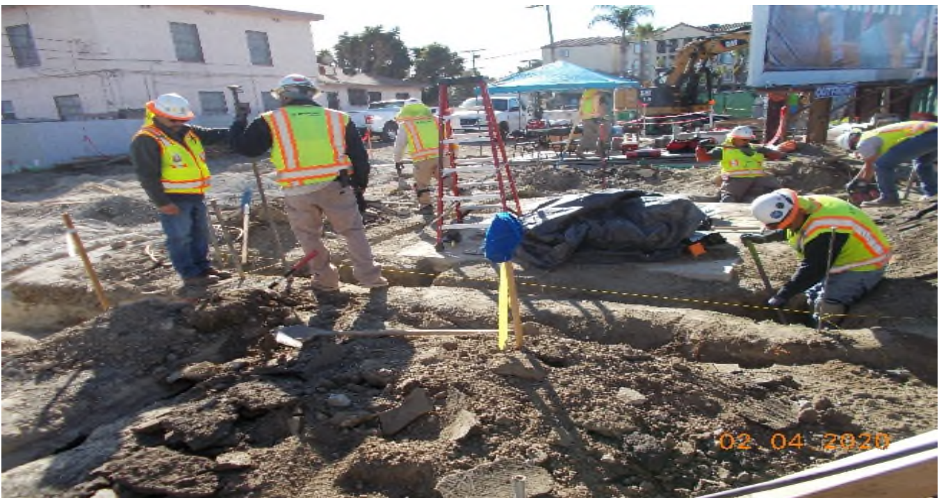
Park Mesa – Excavating trench to continue TPSS#7 ground grid system work on 60th St & Crenshaw Blvd.
