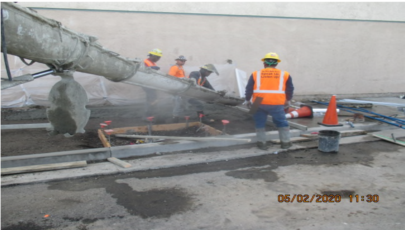
UG3 – Installing block-out forms for curb/tree wells and placing concrete on the eastbound “New Road” sidewalk. 2/5/20
