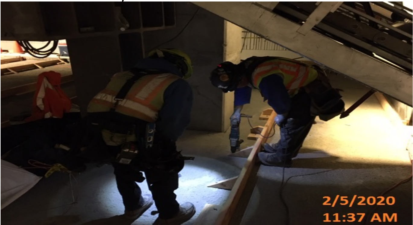
MLK STATION – Continued building formwork for the architectural topping slab at the platform level.
