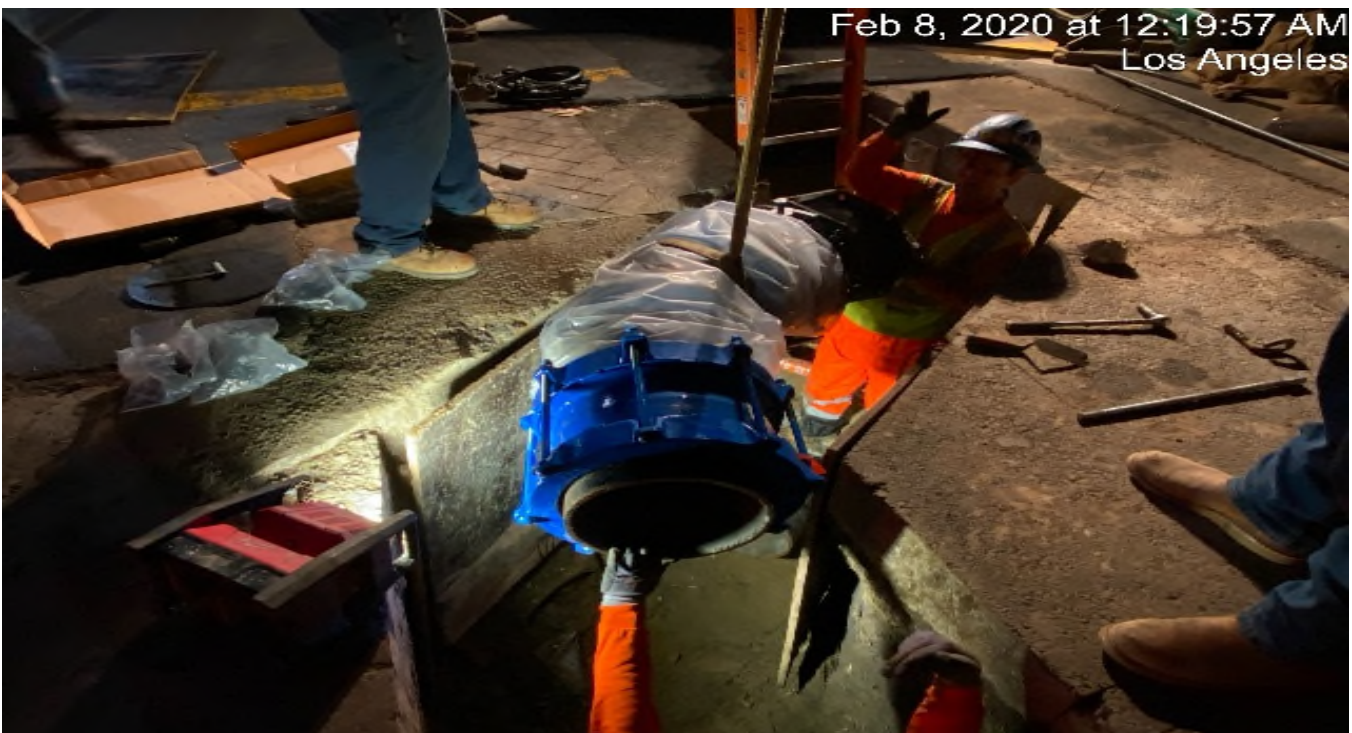
Park Mesa – Continued LADWP main line tie-in at the intersection of 60th St & Crenshaw Blvd.
