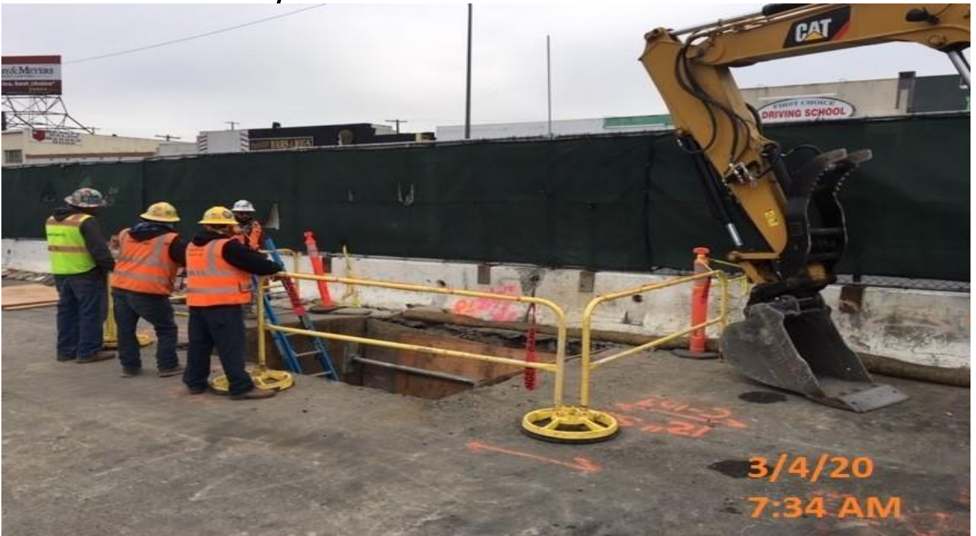
MLK STATION – WSCC crew and Norcal continue exploratory work on leak repair.
