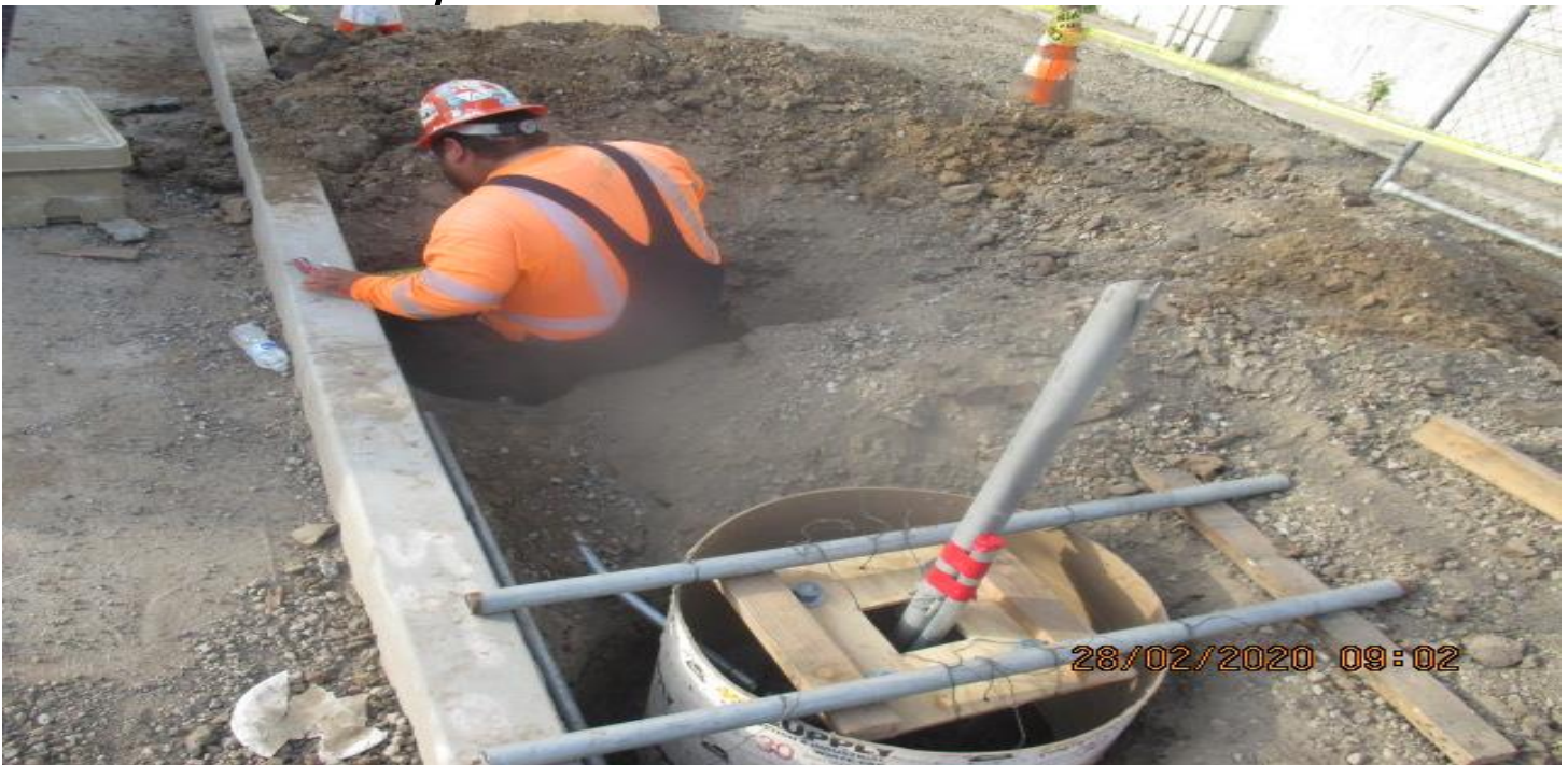
UG3 – Continue installing conduit and pull boxes for street lighting on the north side of the Cul-de-sac radius at North Victoria Ave. 2/28/20
