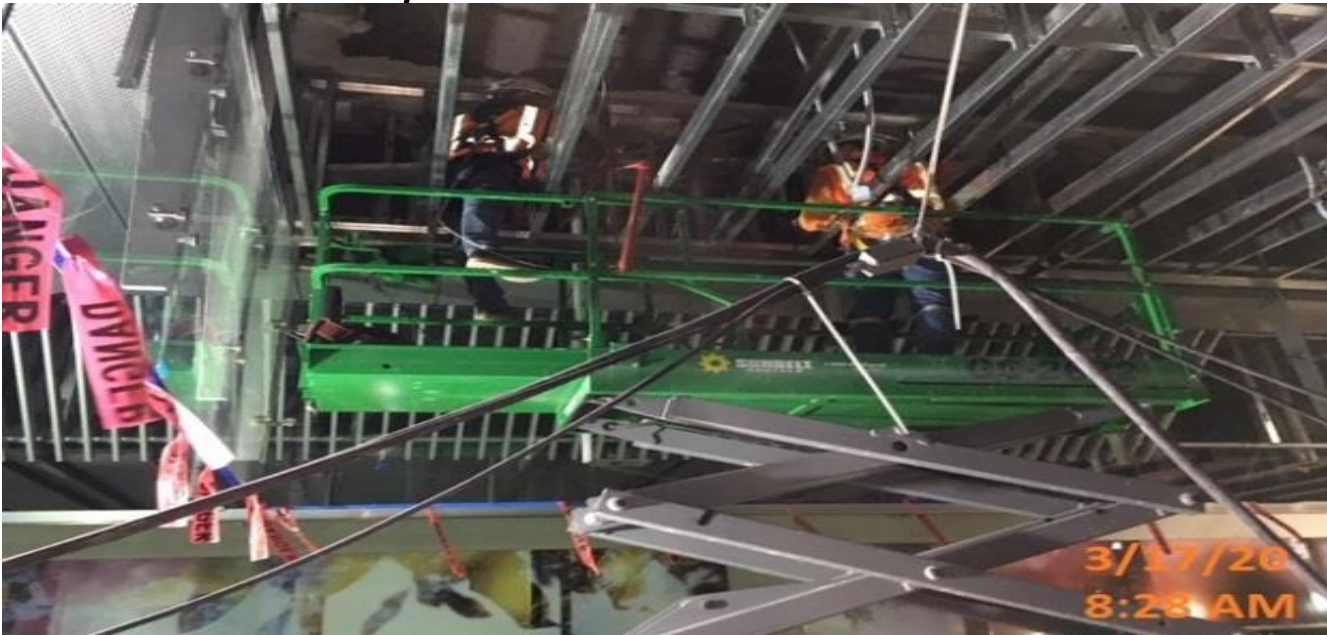
LEIMERT PARK STATION – Installing stainless steel cladding panels on the platform ceiling level.
