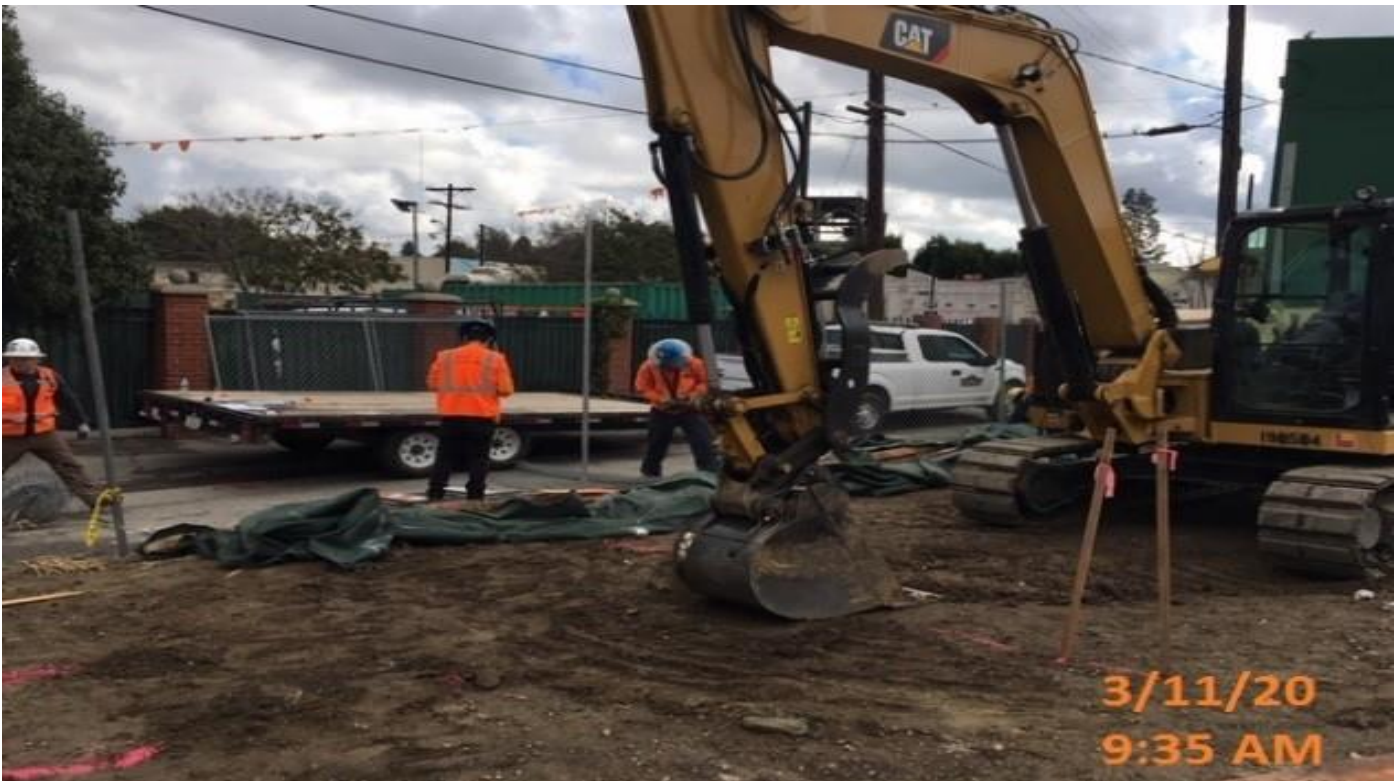
MLK STATION - WSCC removing fencing and placing temp fence prior to excavating for east entrance stairs.
