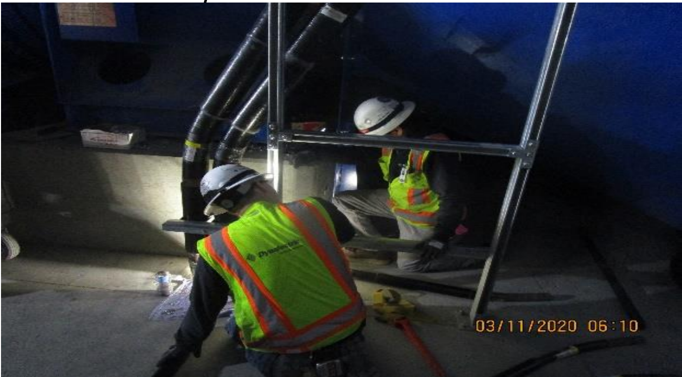
LEIMERT PARK STATION – Continue installing fire rated conduit to the pull box for EVF-6-301 in the South Fan Room C – 102 of the concourse level.
