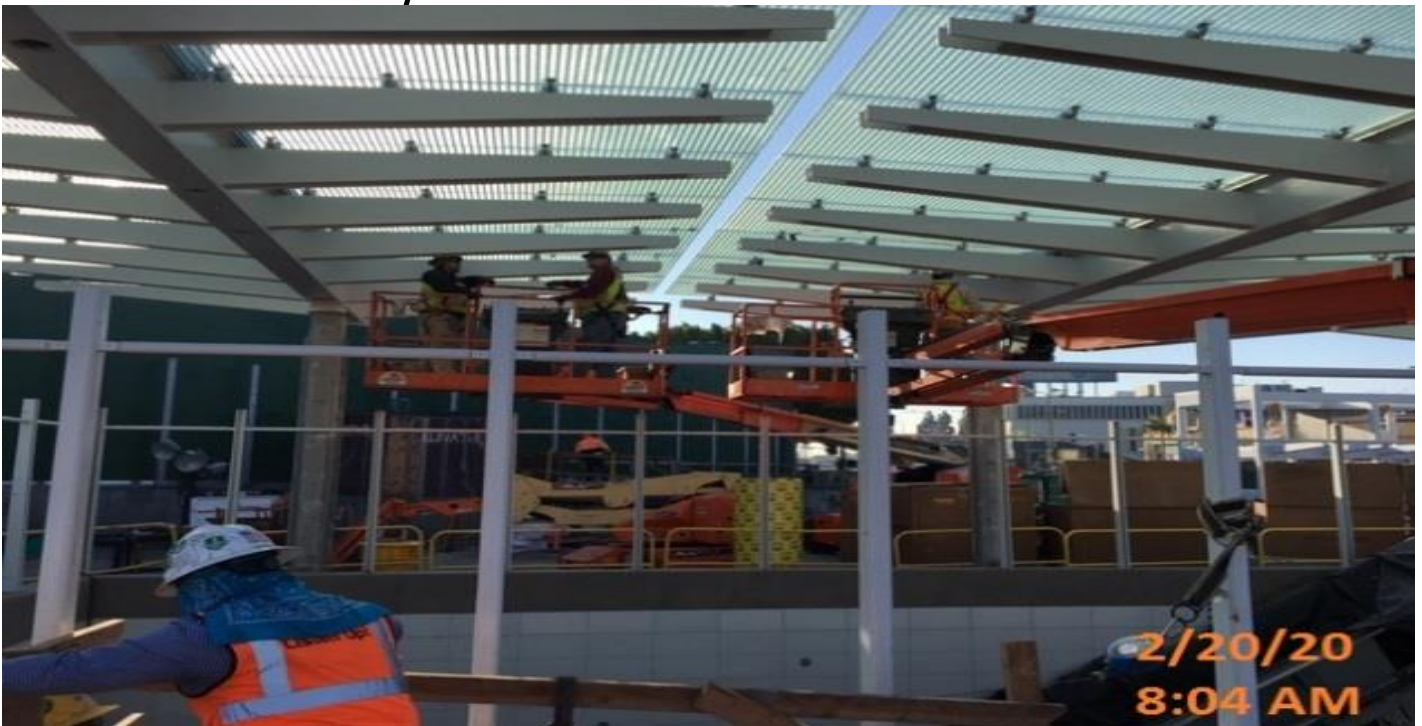
LEIMERT PARK STATION – Continue glass panel installation above the main entrance canopy structure at the plaza level.
