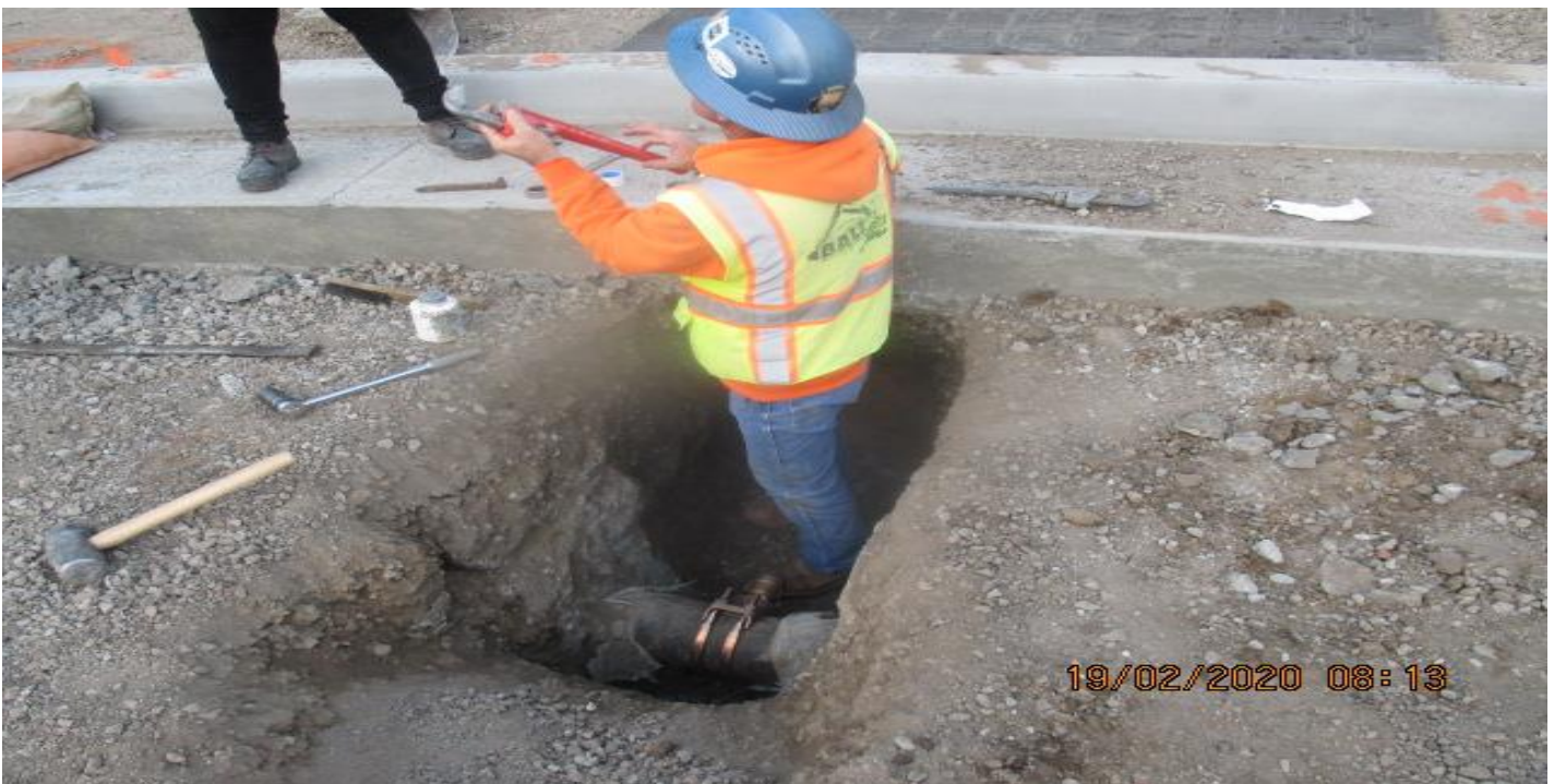
UG3 – Installing new 1” water service pipe line on the new Cul-de-sac radius at North Victoria Ave. 2/19/20
