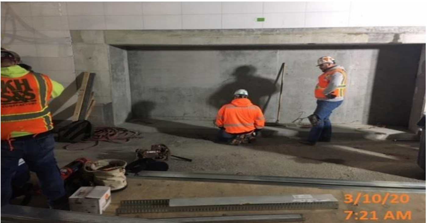
MLK STATION - Installing steel stud track for the ticket vending machine at the concourse level.
