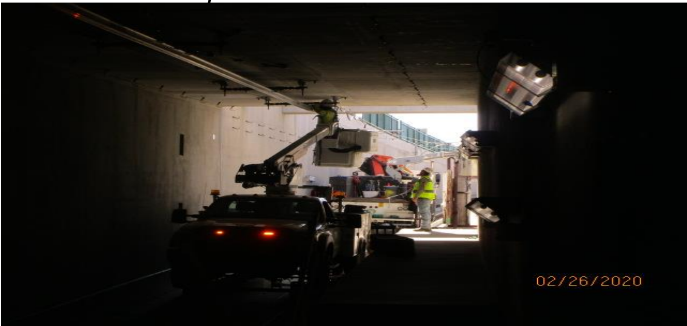
UG4 – Registering and staggering guide sections for the overhead contact rails at the south end portal.
