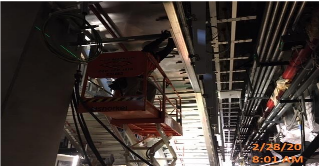
MLK STATION – Continue installation of laminated cladding frame for the metal panels beneath staircase 3 at the platform level.
