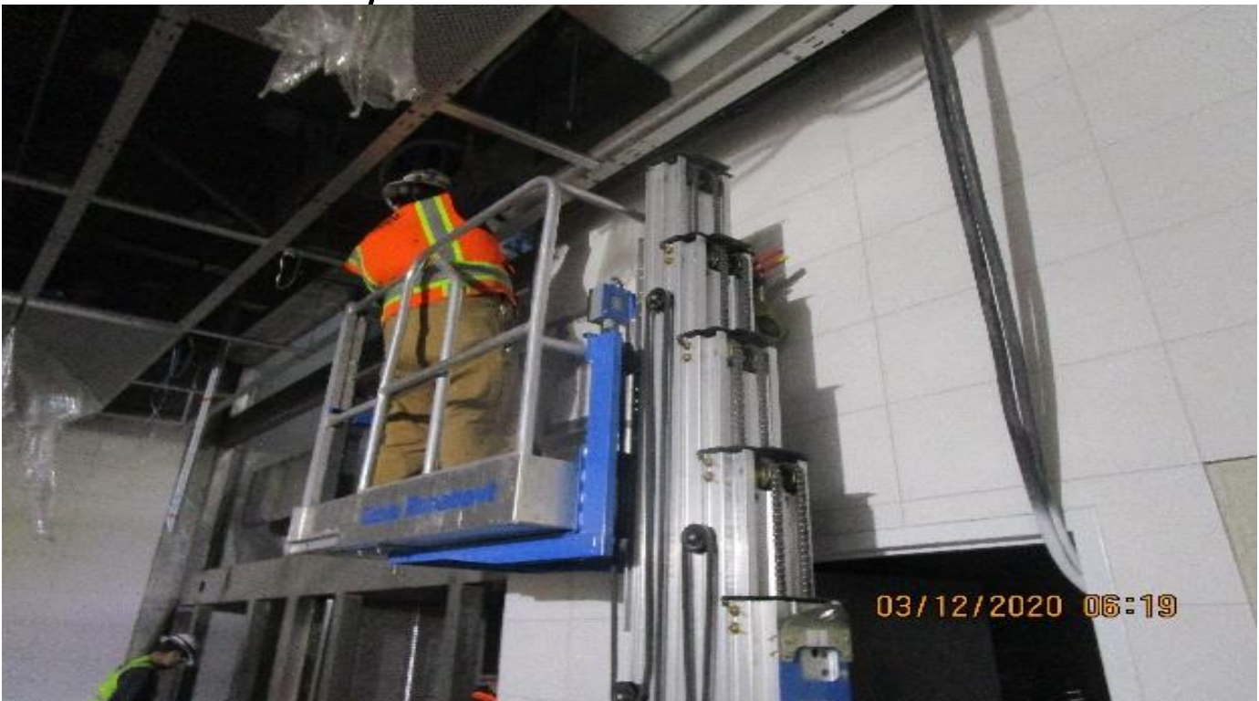
LEIMERT PARK STATION – Continued installing light cove and ceiling panels throughout the Free & Paid Area of the concourse level.
