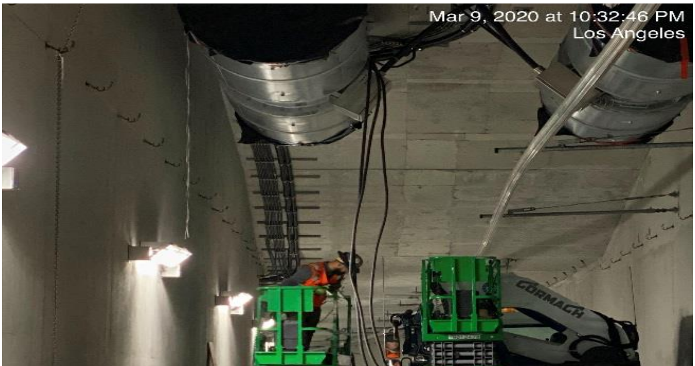
UG-4- – Continue wiring and running cable for the booster fans in the northbound tunnel at Sta 378+75.
