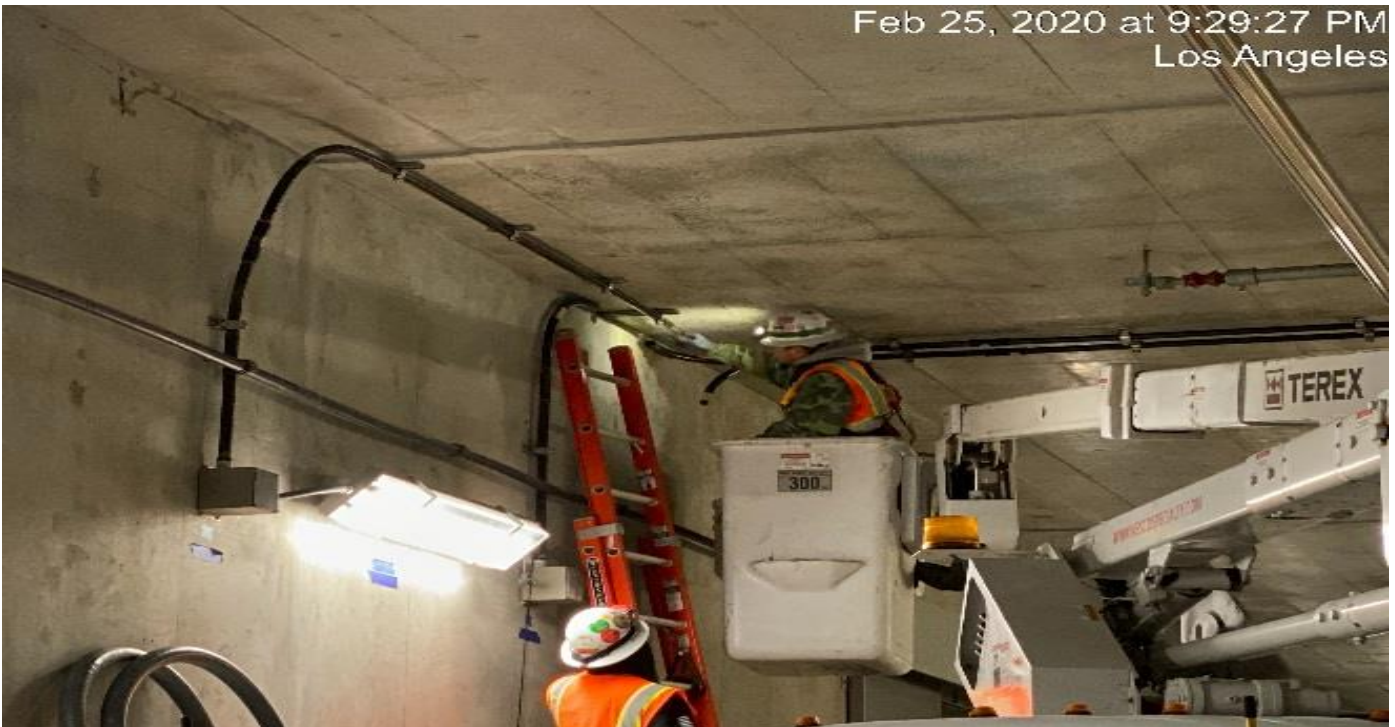
UG3 – Continue installing phenolic conduit for the emergency lighting along the northbound tunnel at Sta 298+00.
