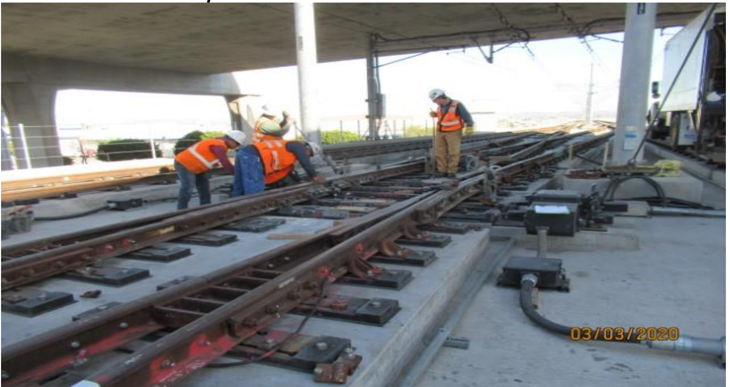
GUIDEWAY - HCC raising rails on MPF for repair work on concrete slab at GL Wye.
