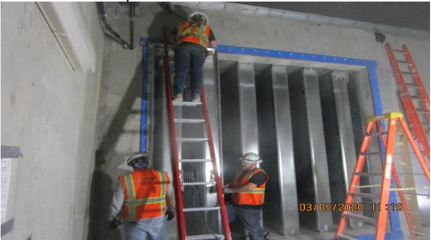
MLK STATION - Installing bird protection screens on the sound attenuators for EVF-7-322 in the North Fan Room C – 142 of the concourse level.
