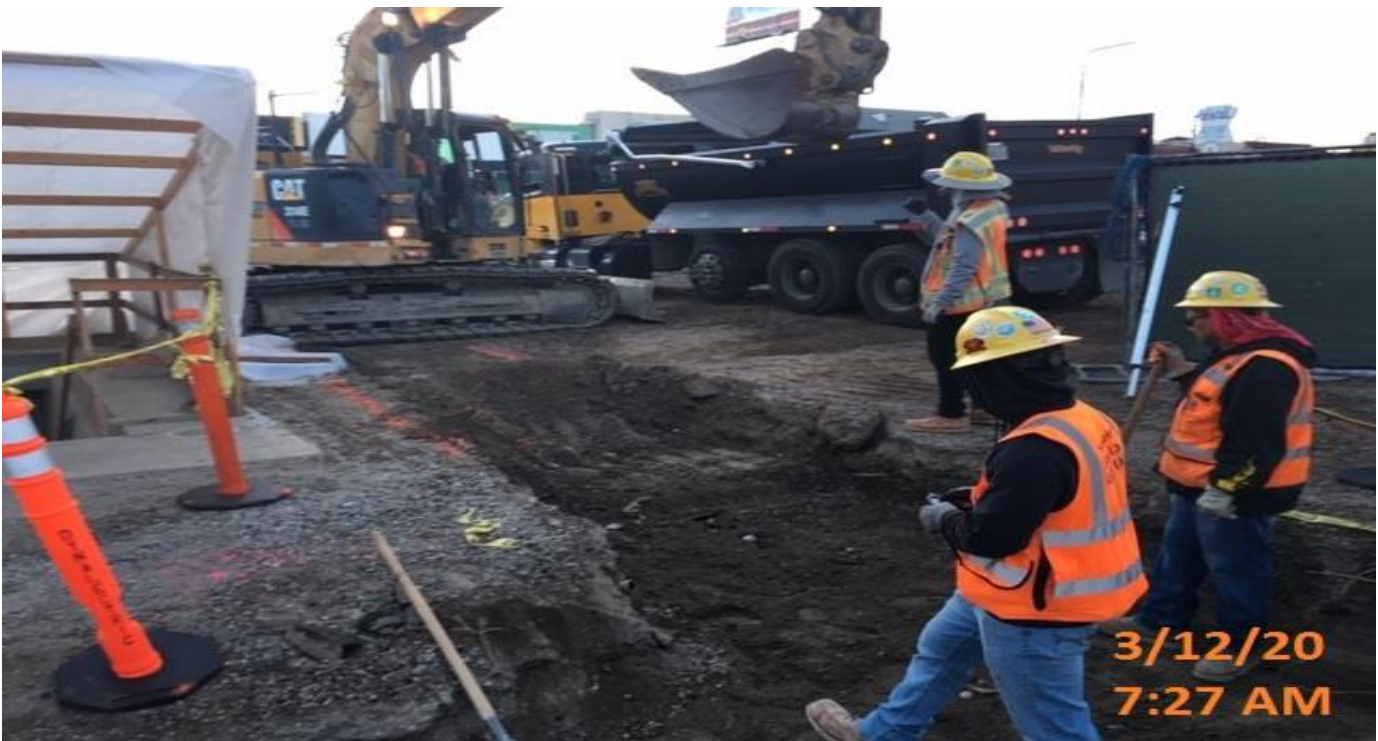
MLK STATION - Continue excavating/demolishing for planter wall footings at the plaza level.
