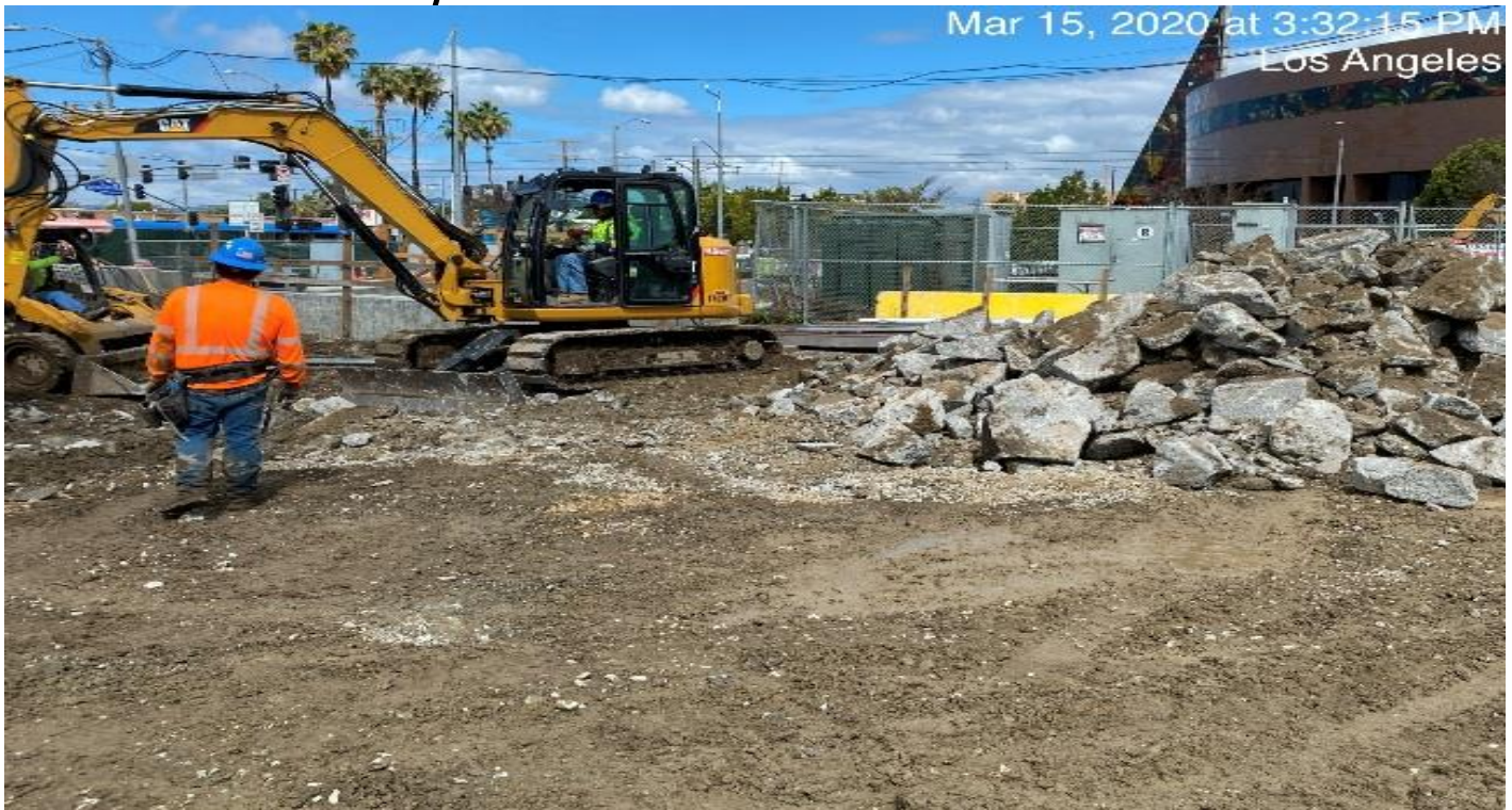
EXPO STATION- Continue demolition/excavation of concrete slabs east of the plaza in preparation for trenching and underground electrical fiber rough in.
