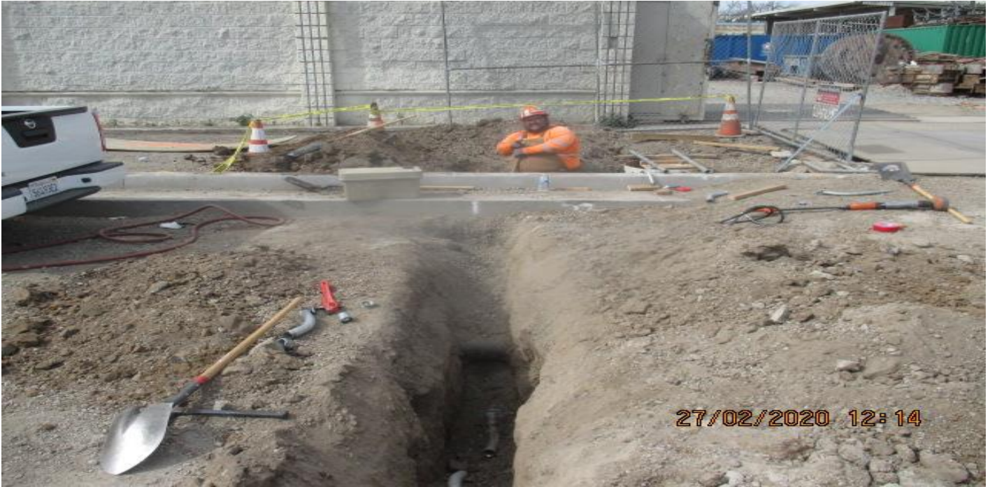
UG3 –Installing conduit and pull boxes for street lighting on the north side of the Cul-de-sac radius at North Victoria Ave. 2/27/20
