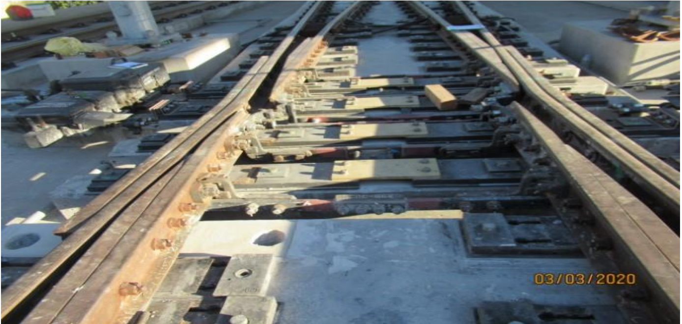
GUIDEWAY - MPF at GL Wye STA 13+90 incomplete work on concrete.
