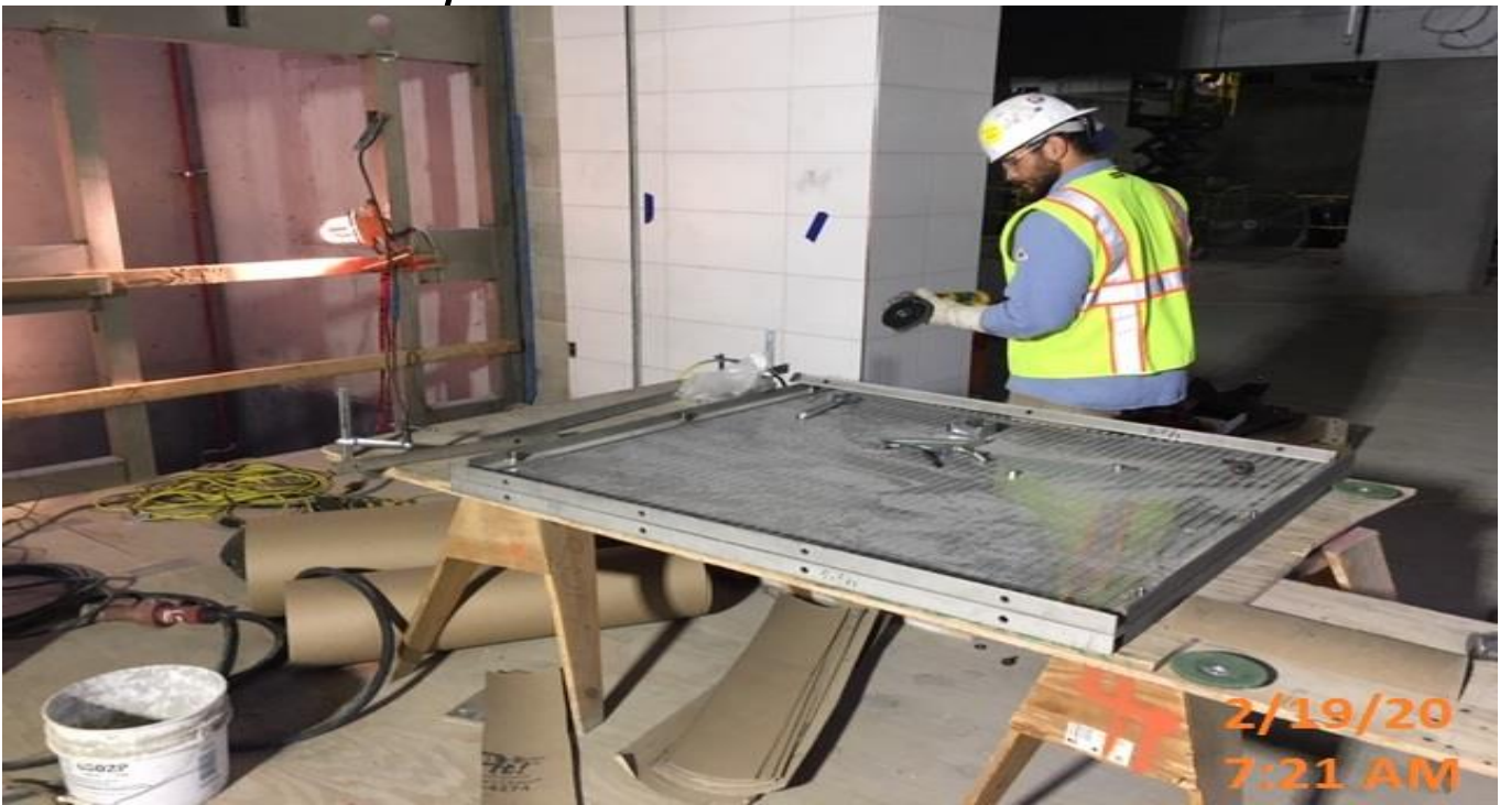
EXPO STATION – Installing divider screens to Elevator shaft/pit 1&2 at the concourse level.
