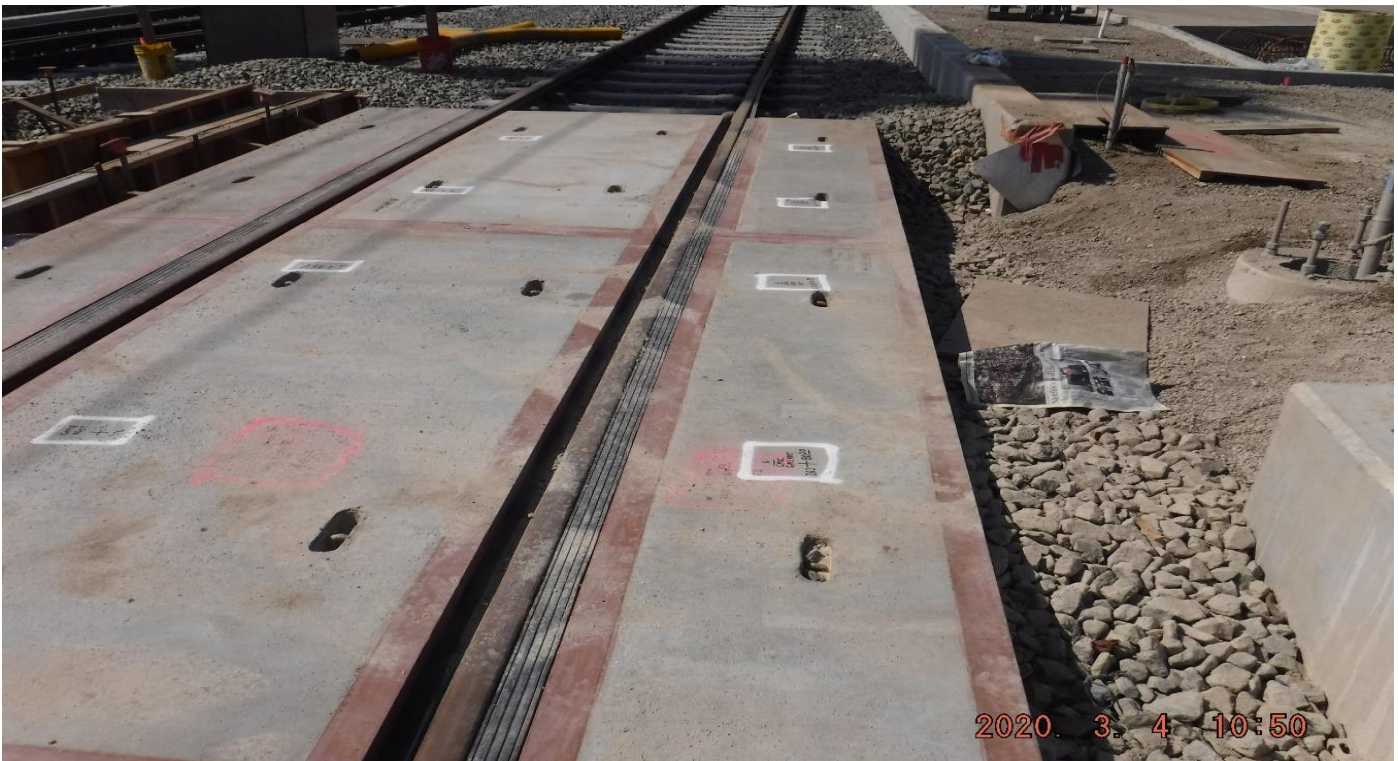
WEST Blvd - STA262+74_ Looking South_ Dirt spilled over TK ballast_ PUNCH LIST_ West.
