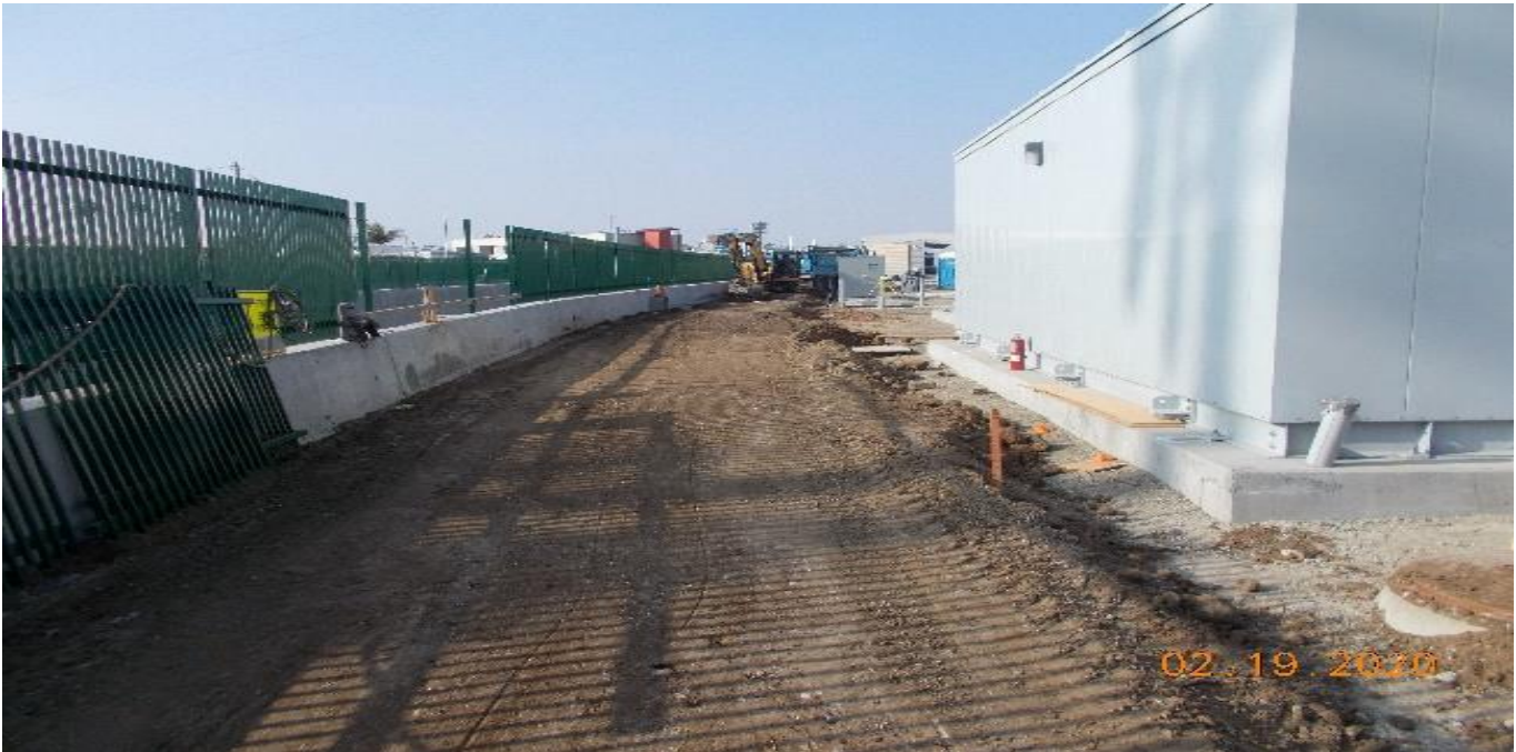
UG3 – Excavating/grading around the auxiliary power site at Victoria Yard adjacent to the south end portal.
