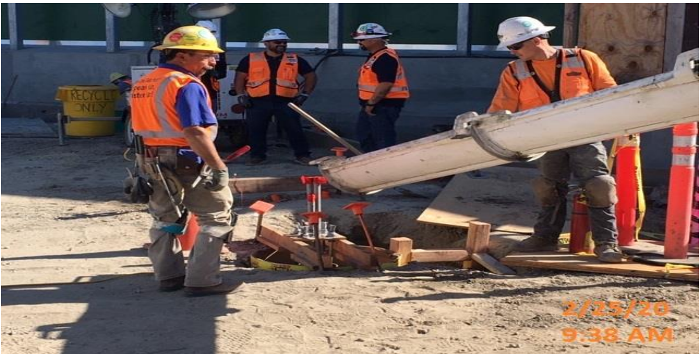
LEIMERT PARK STATION – Began perimeter formwork for slab encasement of irrigation lines for the main entrance canopy at the plaza level.
