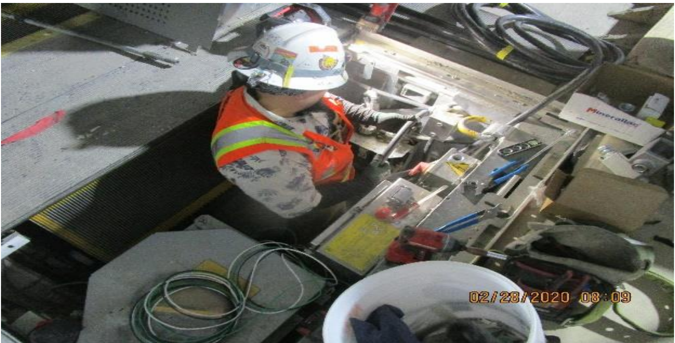
LEIMERT PARK STATION – Installing conduit to junction boxes for Escalators 3&4 at the intermediate level.
