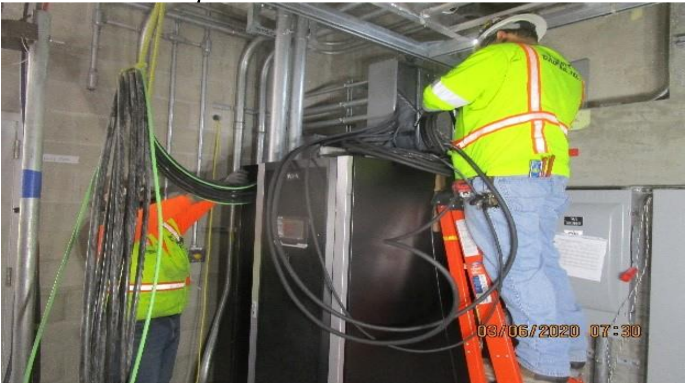
Crenshaw/Vernon – Vernon, TC&C C112, begin pulling 3.0 feeders & #4 ground from comm UPS to battery`s at battery room C113.
