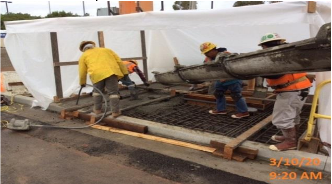
MLK STATION - Began placing concrete on top of the fire protection valve pit access hatch at the plaza level.
