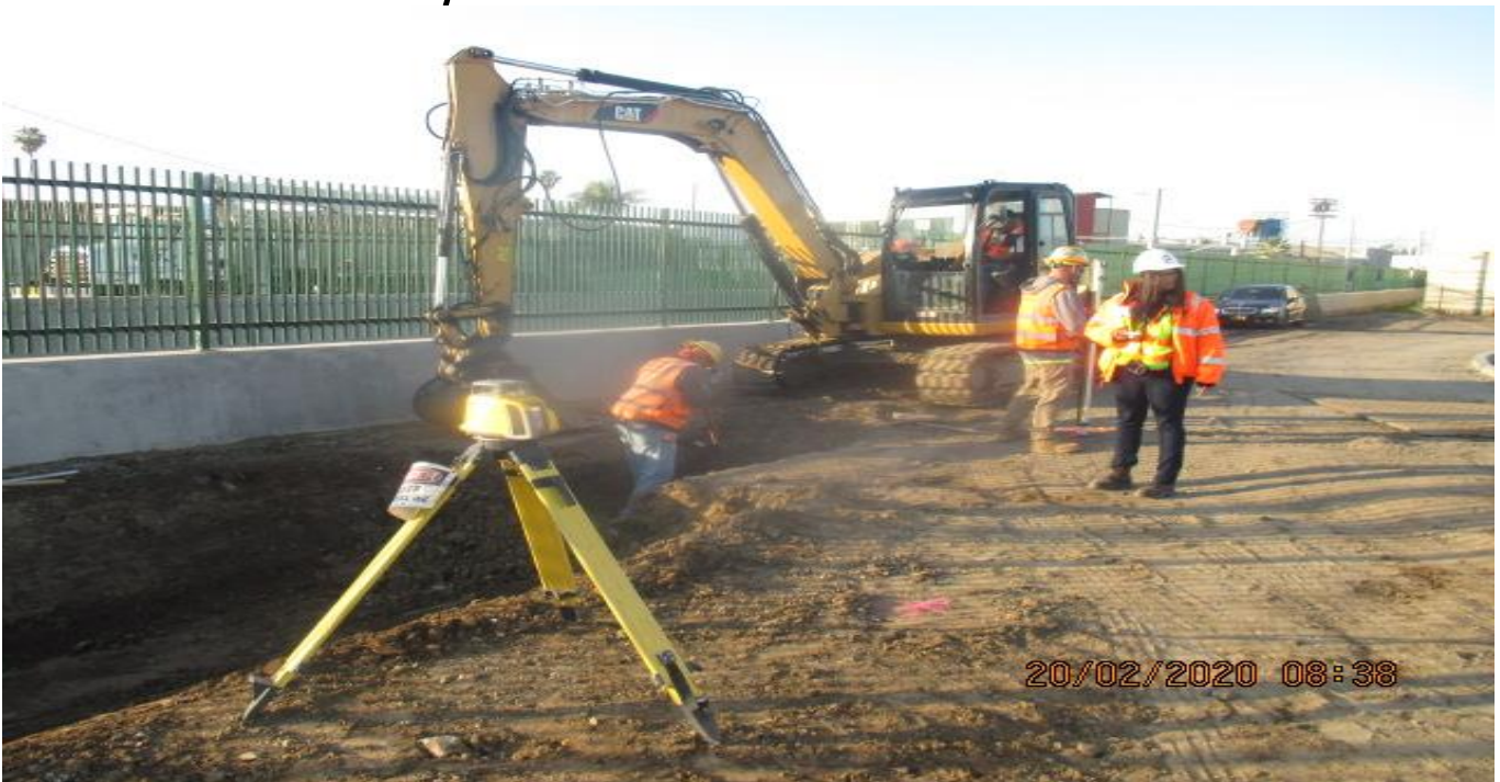
UG3 – Continue excavation for culvert drainage along the southbound barrier wall from Sta 279+20 – 282+93. 2/20/20
