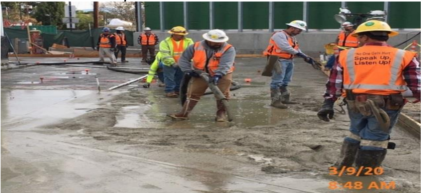
LEIMERT PARK STATION – Placing slurry at the south end of the main staircases of the plaza level.
