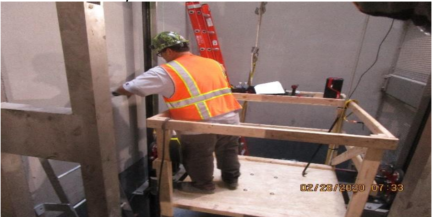
LEIMERT PARK STATION – Continue guide rail bracket support for Elevator hoist way/pit 2 at the concourse level.
