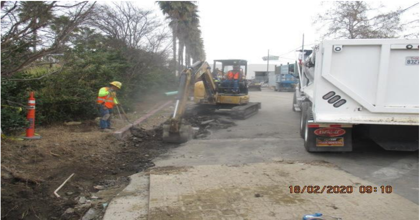
EXPO STATION – Continue demolition/excavation of both roadway shoulders for new Cul-de-sac entrance on Bronson St. east of the plaza. 2/18/20
