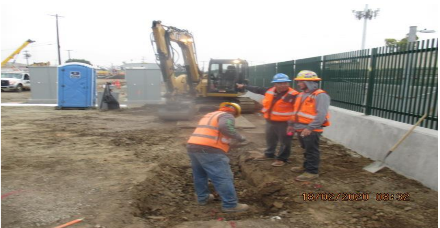
UG3 – Continued excavation/compaction of the new Cul-de-sac in preparation for curb/gutter installation and concrete placement at North Victoria Ave. 2/4/20
