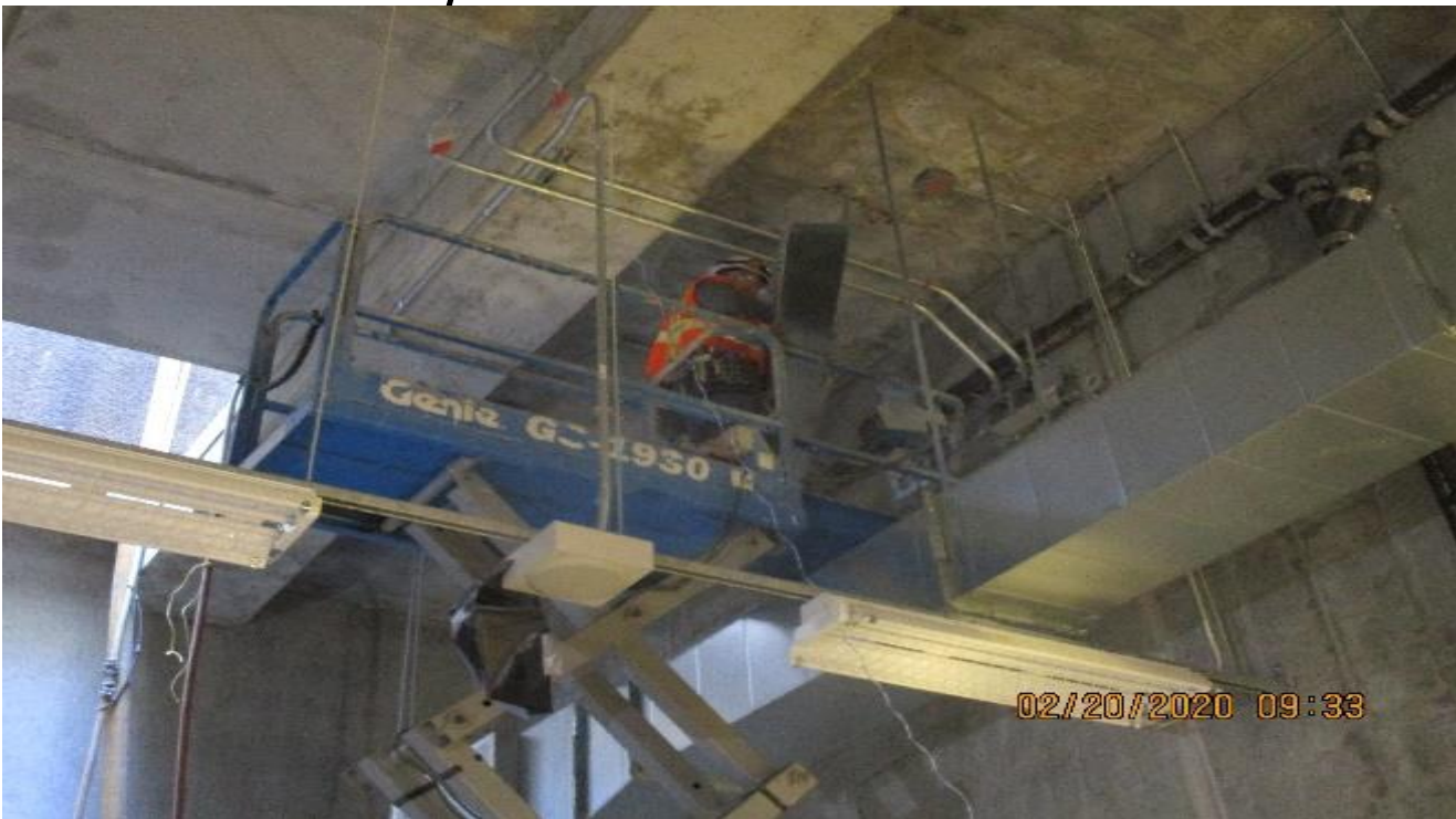
MLK STATION – Continue installing sheet metal drip pans for the overhead drainage in TPPS Room T109 of the invert level.
