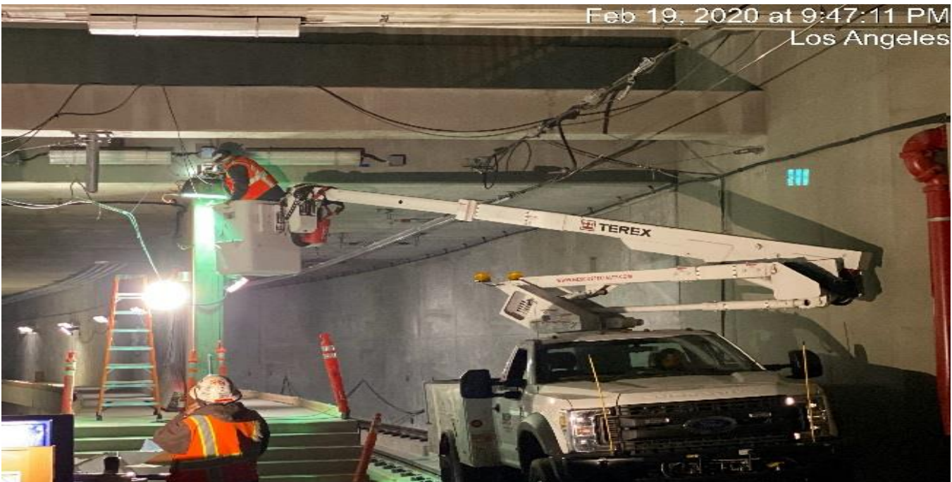
UG3 – Continue pulling wire for the emergency lighting at the south end portal entrance.
