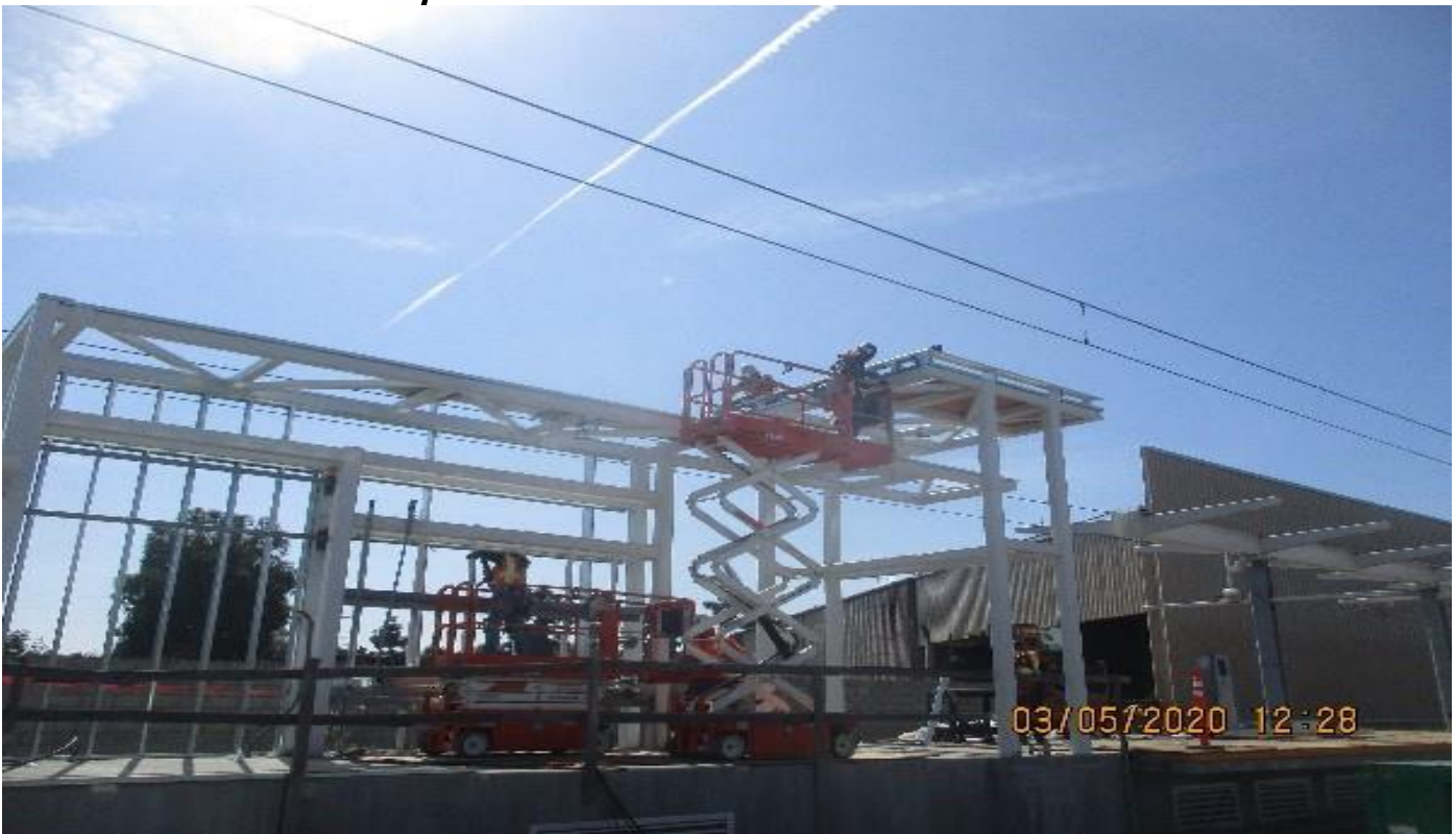
WEST Blvd - KHS&S place rail and roof panels at West Sta ticket pavillians.
