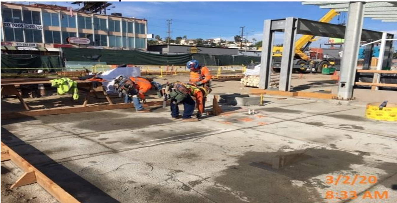
LEIMERT PARK STATION – Marking gridlines in preparation for the architectural topping slab at the plaza level.
