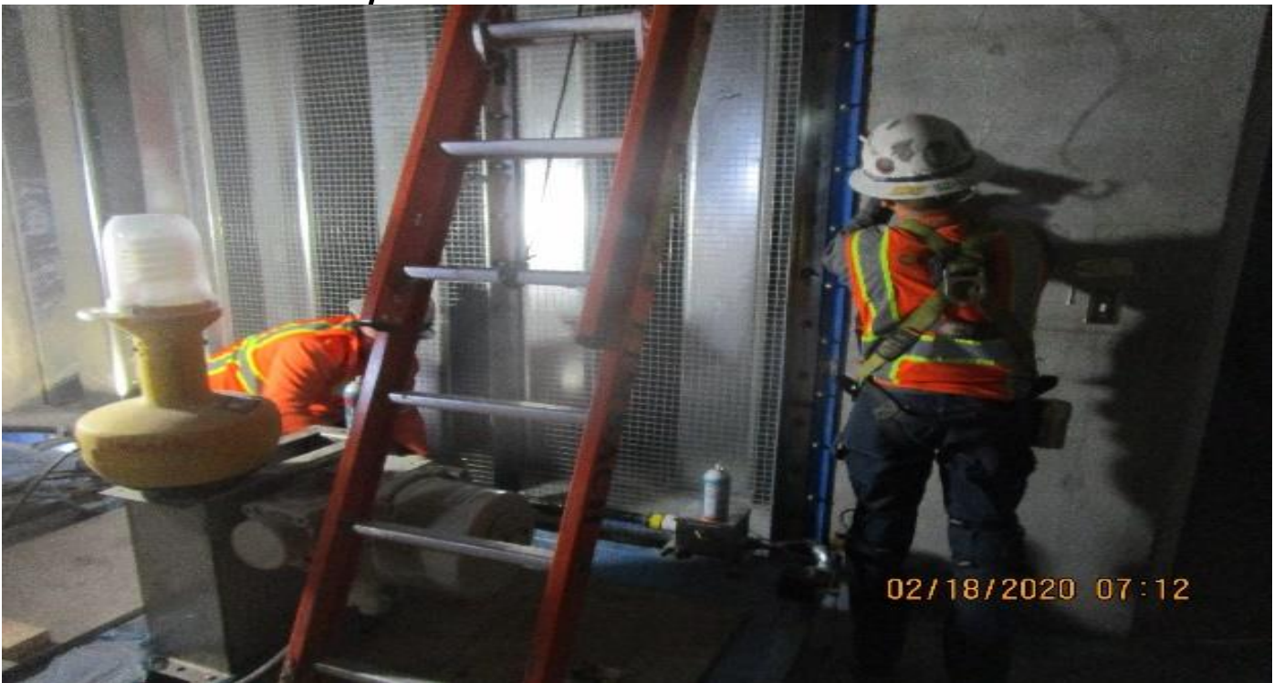
LEIMERT PARK STATION – Installing bird protection screens on the sound attenuators in both the North C – 126 and South C – 102 Fan Rooms of the concourse level.
