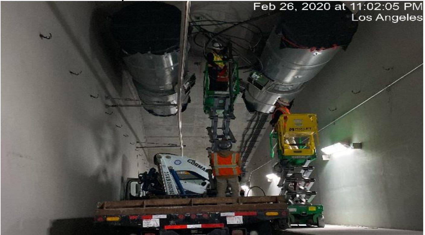
UG4 – Continue wiring and running cable for the booster fans on both north and southbound tunnels.
