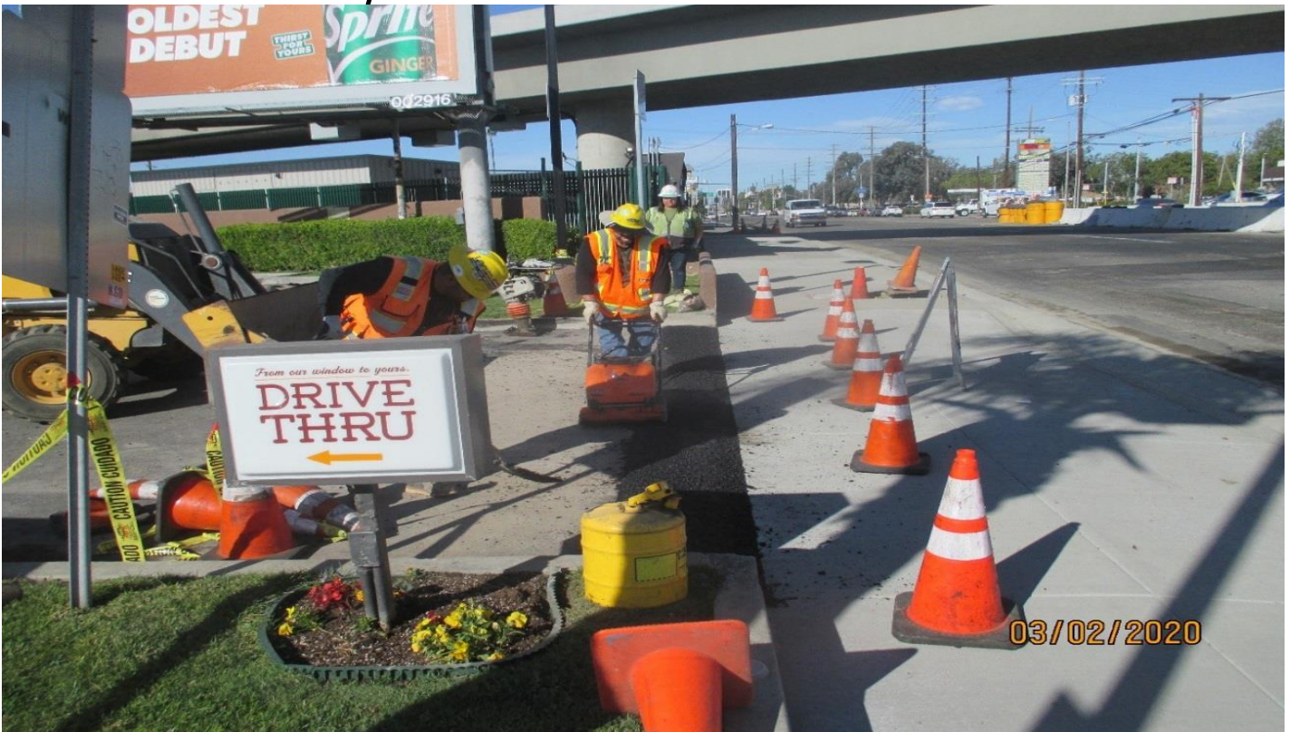
MANCHESTER AVE- Slot paving for the El Pollo Loco driveway on Manchester. Facing west.
