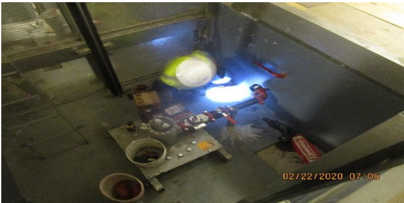
MLK STATION – Installation 3” hydraulic line to valve for Elevator hoist way/pit 3&4 at the platform level.
