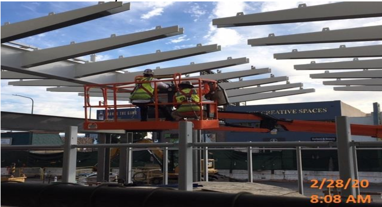
MLK STATION – Began glass panel fitting installation above the main entrance canopy structure at the plaza level.
