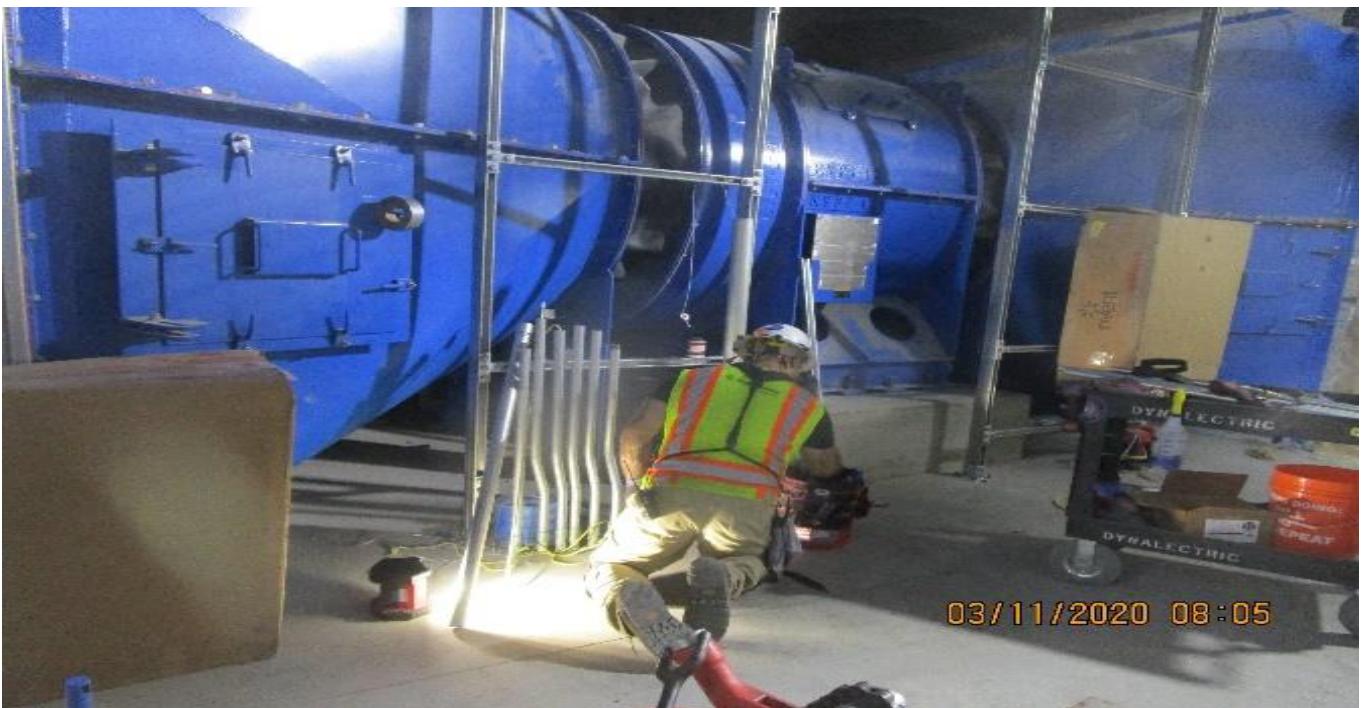
MLK STATION - Began rough in for fire rated conduit installation to the pull box for EVF-7-121 in the South Fan Room C – 102 of the concourse level.
