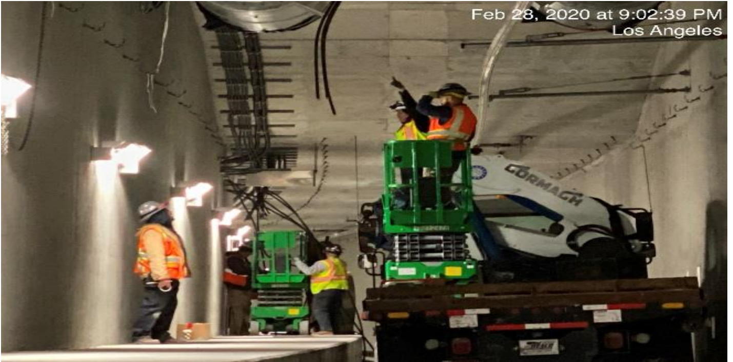
UG4 – Continue wiring and running cable for the booster fans in the northbound tunnel at Sta 376+50.
