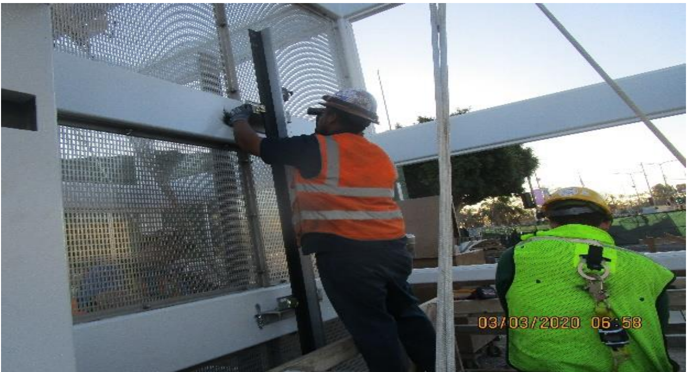
LEIMERT PARK STATION – Continue guide rail bracket support for Elevator hoist way/pit 1 at the plaza level.
