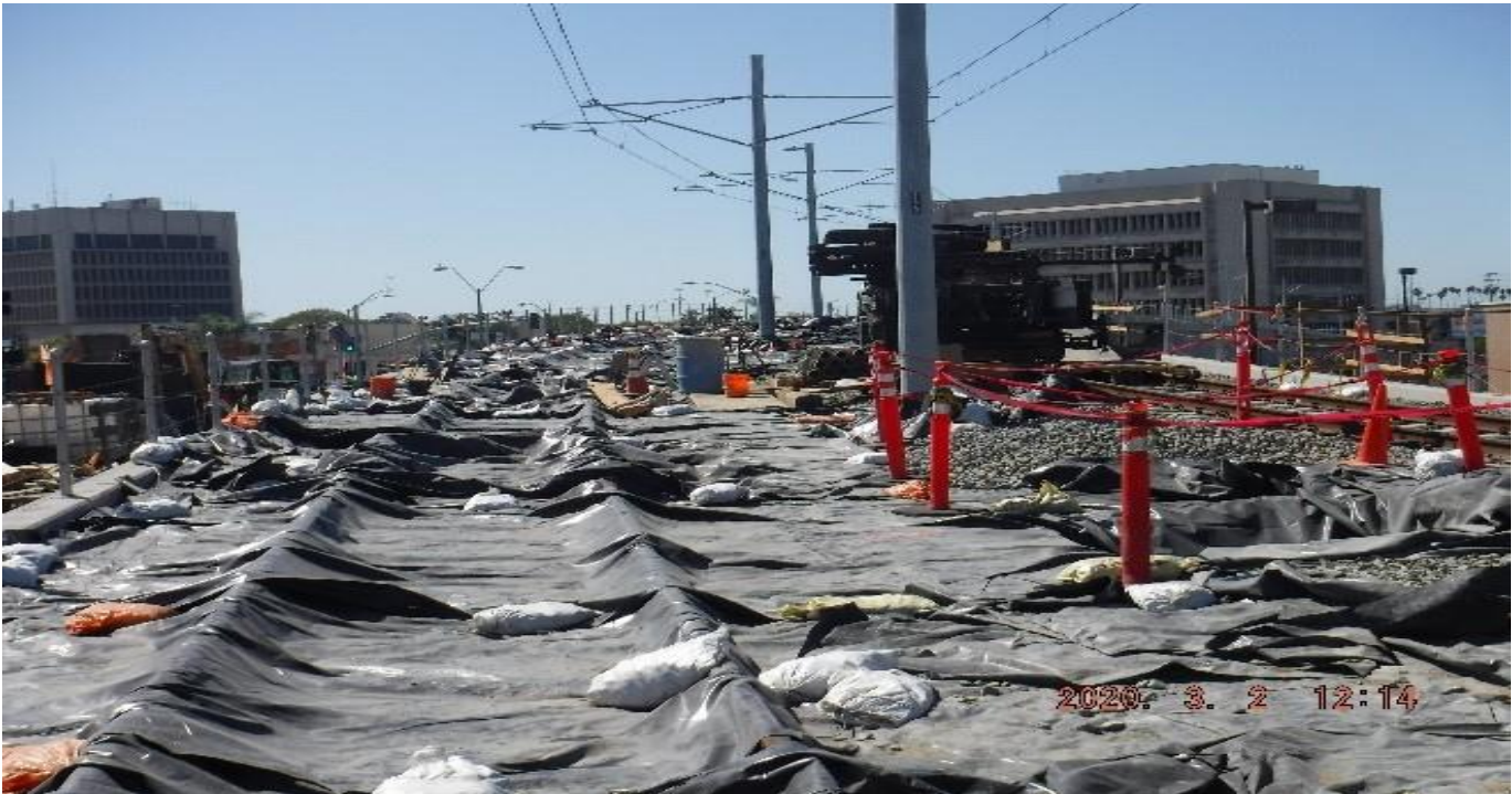
LA BREA – STA 206+00 TK#4-NB looking south – Geotechnical investigation in progress south of La Brea Station.
