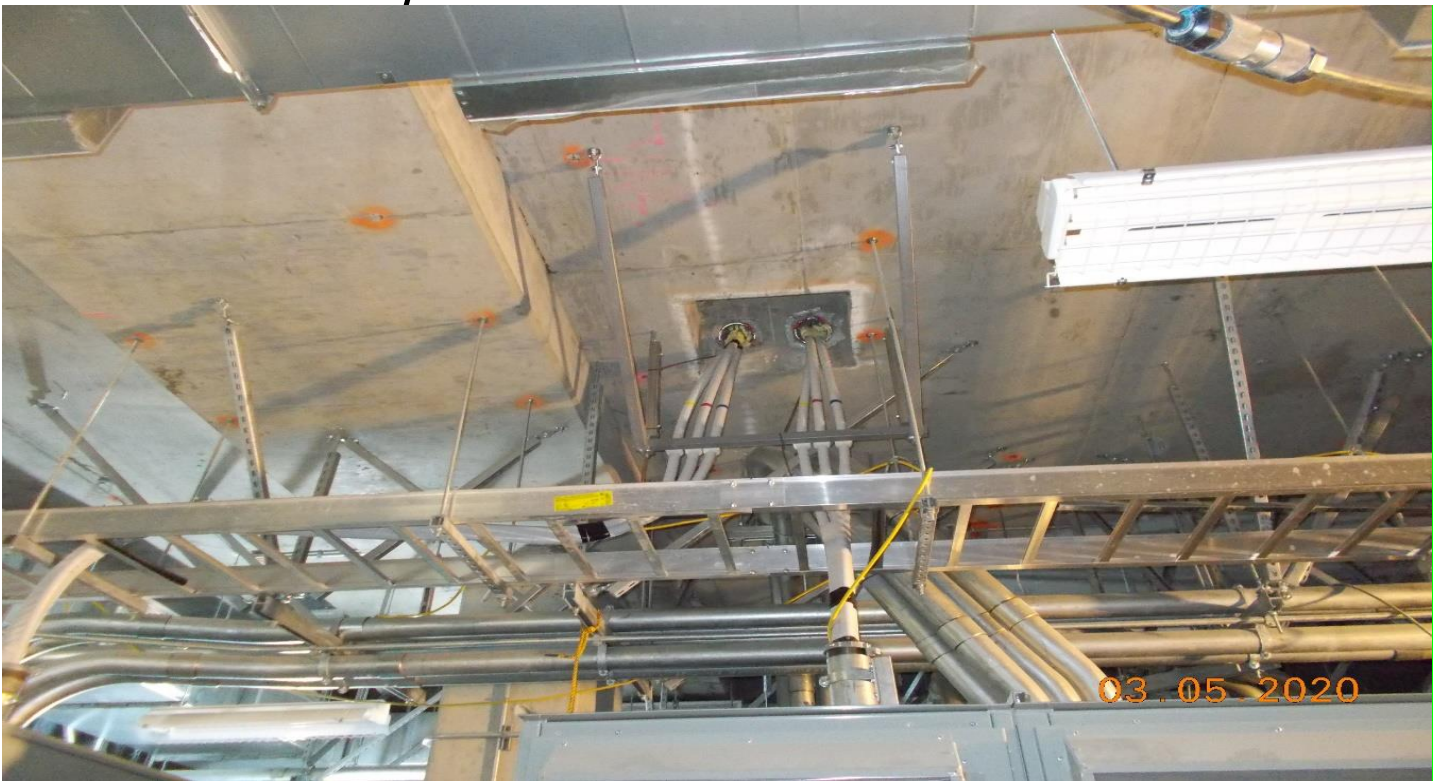
MLK STATION – In Aux Pwr room south Faith Electric had installed a support structure for the high voltage cables.
