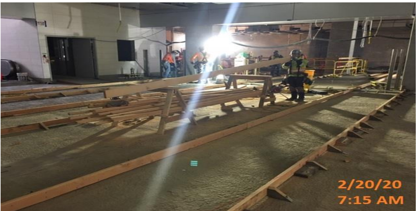
MLK STATION – Continue formwork for the architectural topping slab at the concourse level.
