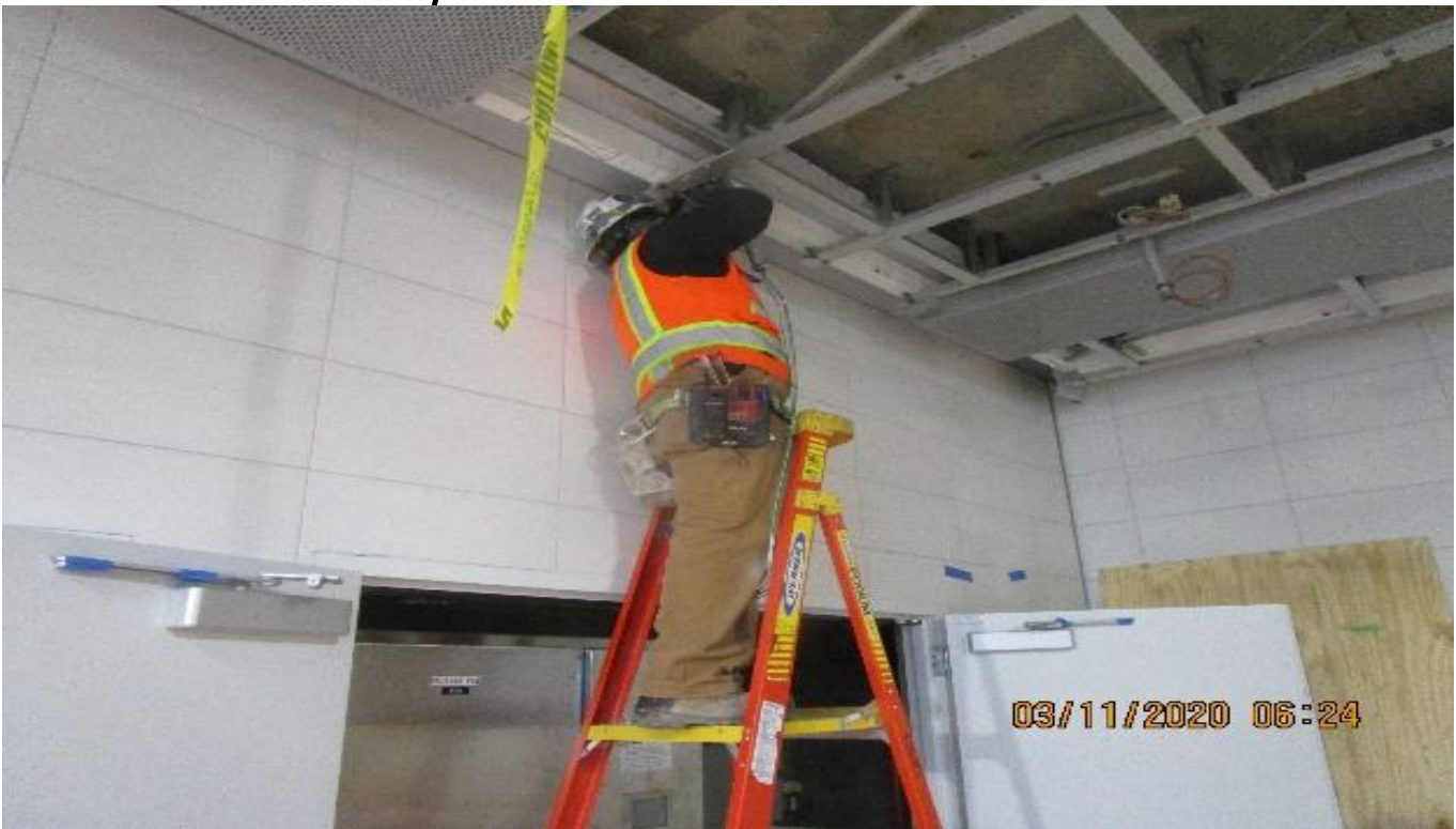
LEIMERT PARK STATION – Installing light cove and ceiling panels at the intermediate landing.
