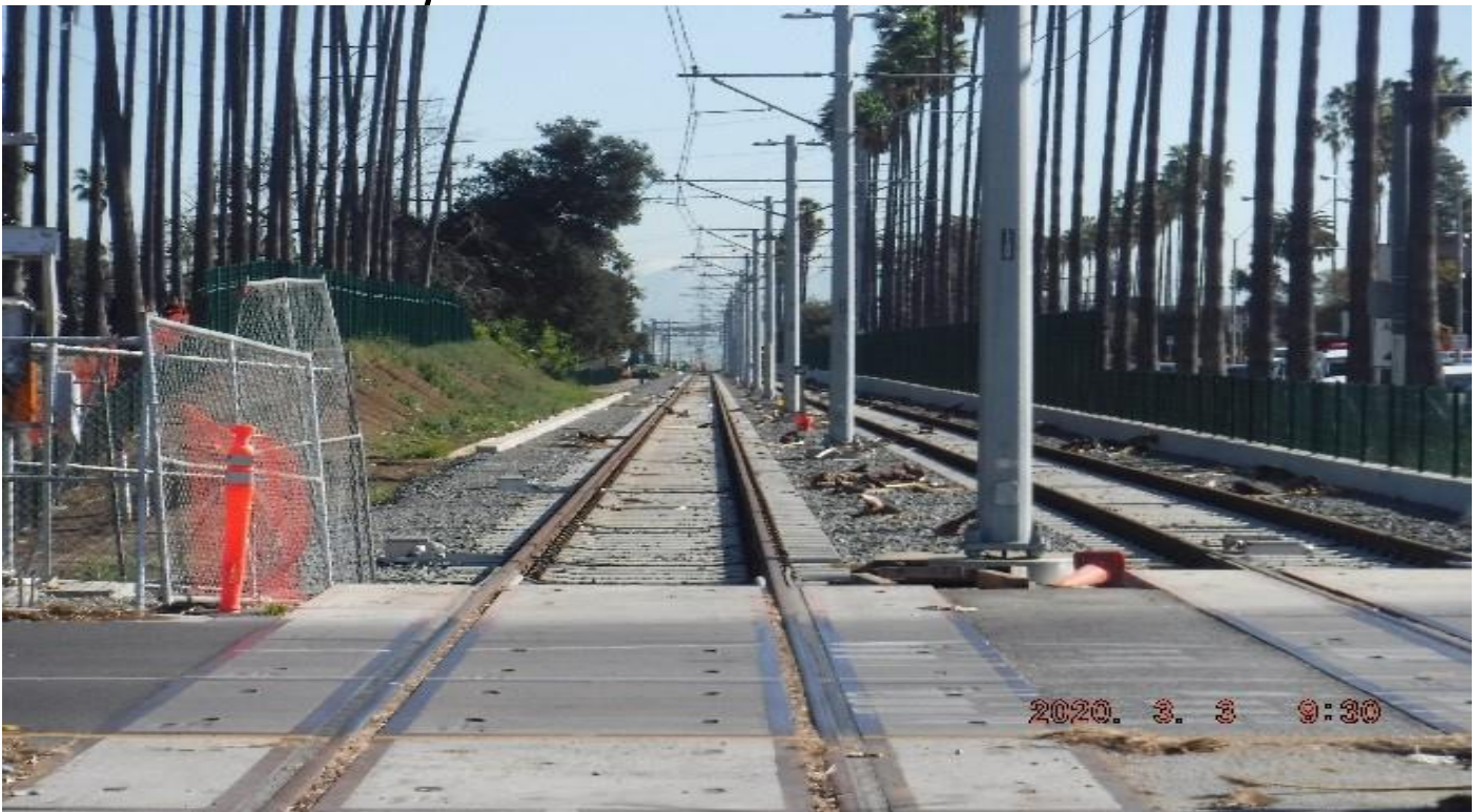
HIGH STREET- STA 225+50 TK#3-SB looking north – no track work north of Centinela Ave; fence work left side R/W.
