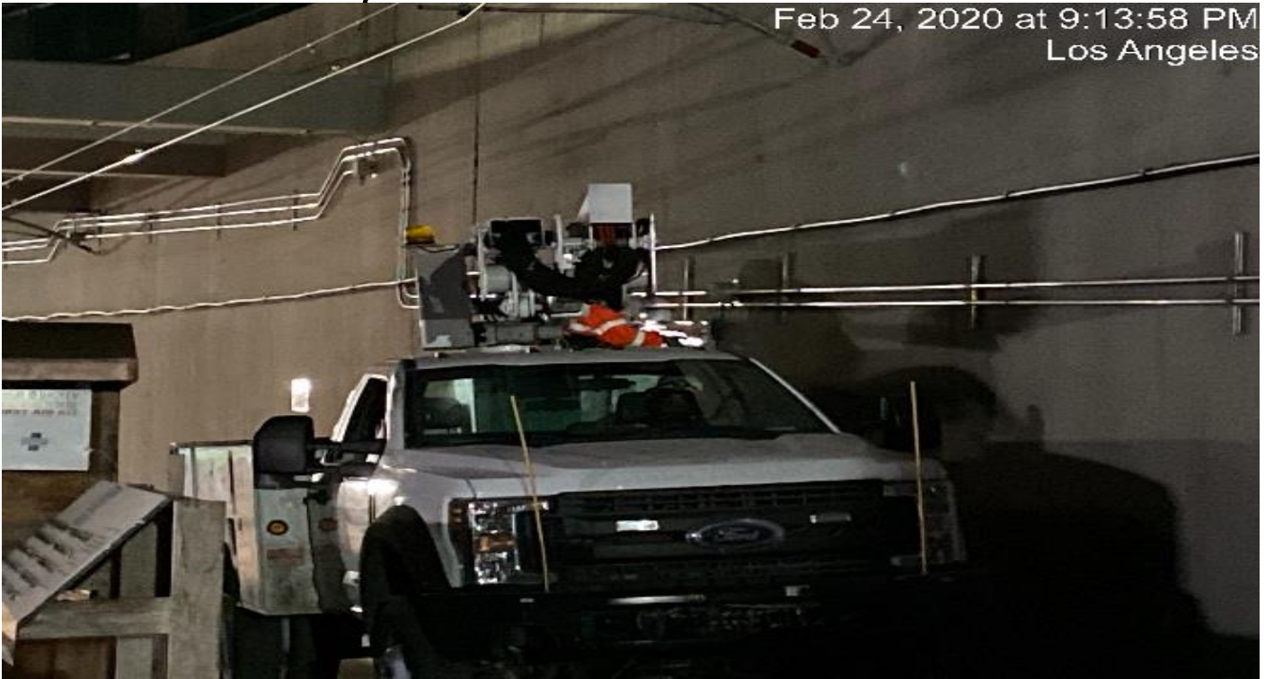
UG3 – Continue pulling wire for the emergency lighting at the south end portal entrance.
