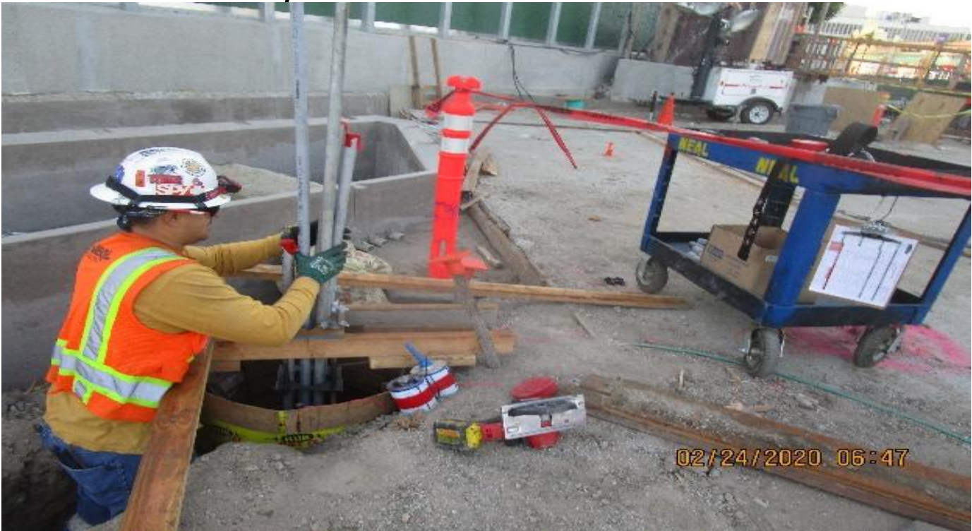
LEIMERT PARK STATION – Setting sonotube foundation forms and rough-in of PVC footings for the installation of the luminaire light posts at the plaza level.
