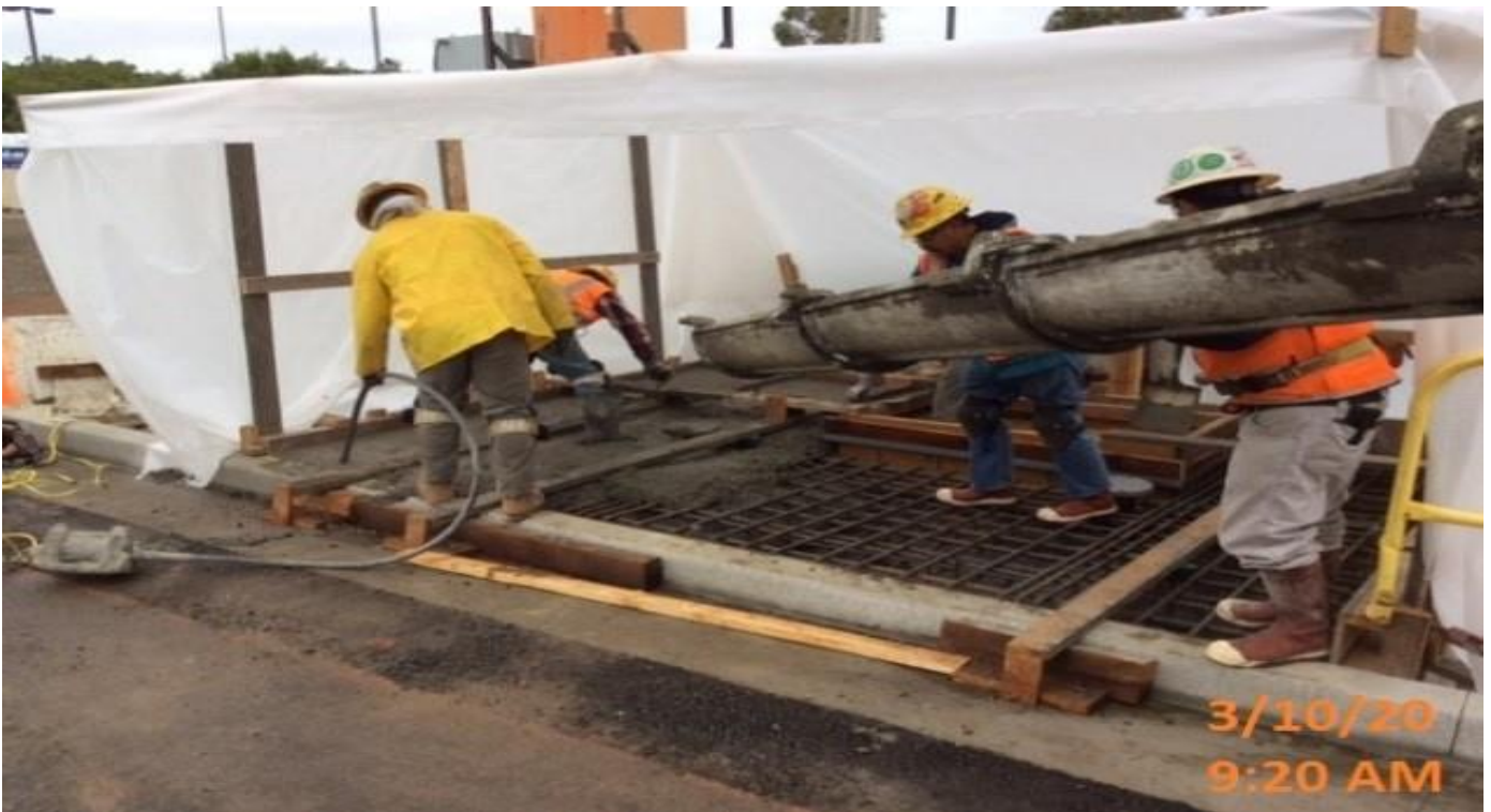
MLK STATION – WSCC crew placing concrete for fire protection valve pit top.
