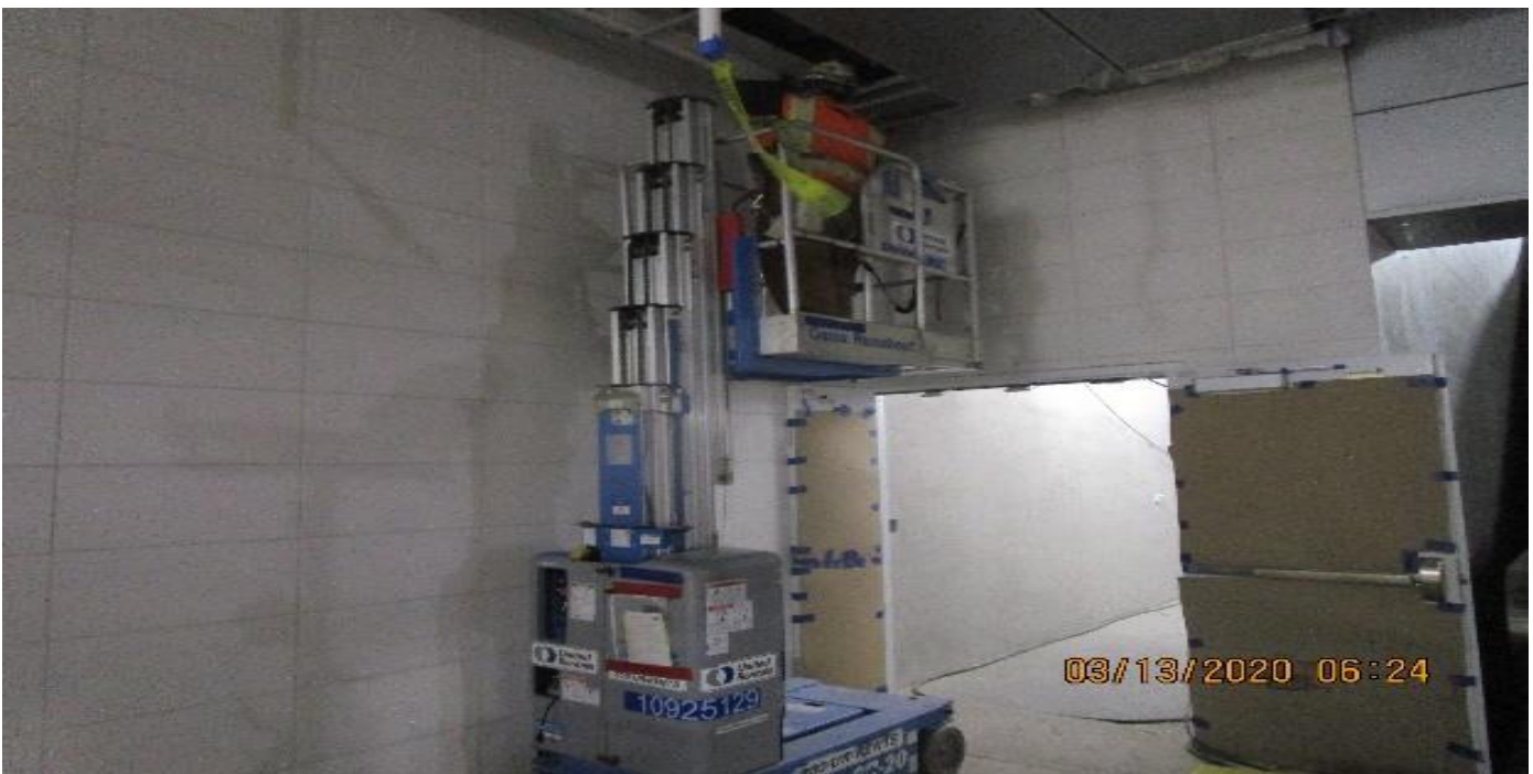
LEIMERT PARK STATION – Continued installing light cove and ceiling panels throughout the Free & Paid Area of the concourse level.
