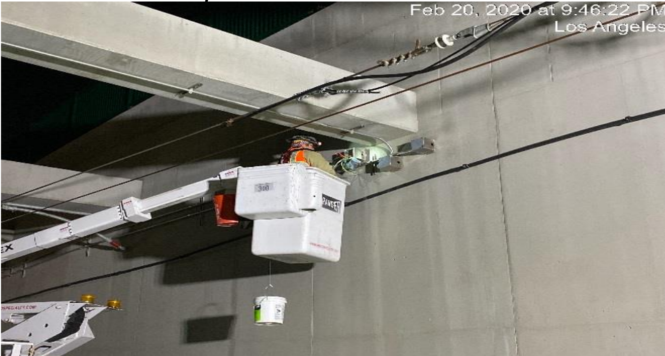
UG3 – Continue pulling wire for the emergency lighting at the south end portal entrance.
