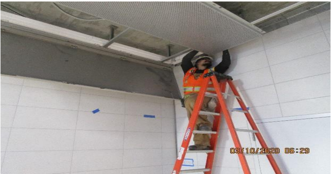
LEIMERT PARK STATION – Installing light cove and ceiling panels at the intermediate landing.
