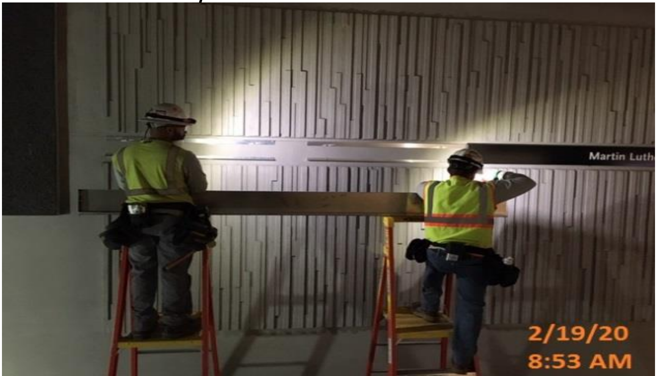
MLK STATION – Continue installing hardware and signage identification along the northbound track of the platform level.
