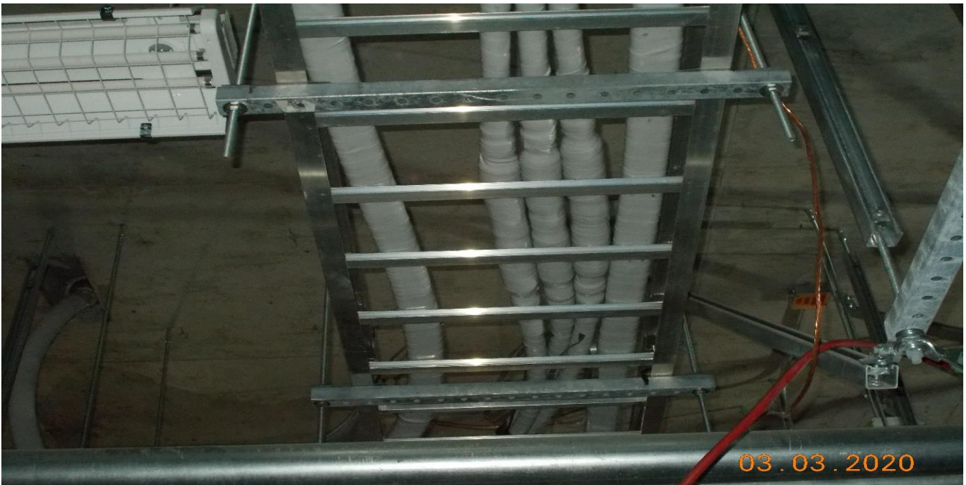
Crenshaw/Vernon – Aux Pwr room south has unterminated high voltage cable grounds in the cable tray.
