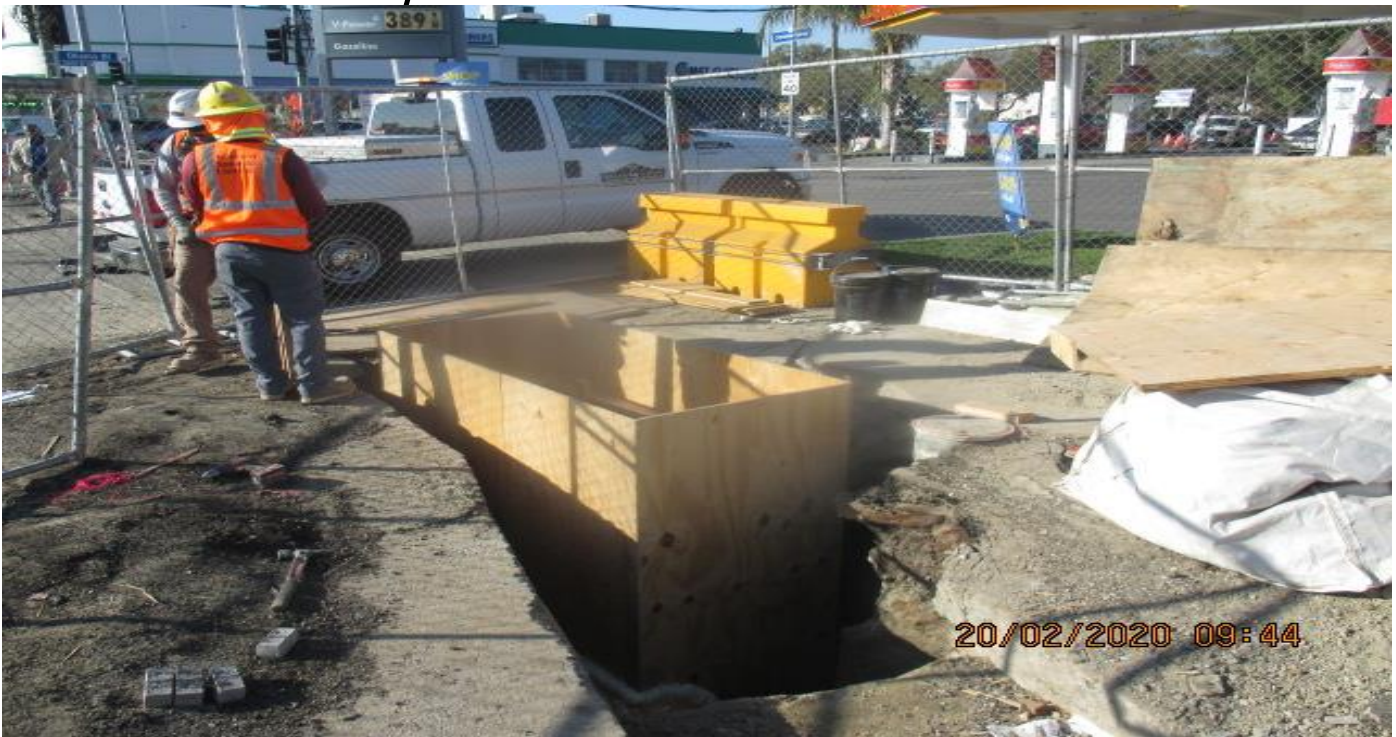
EXPO STATION- Forming and installing rebar for Catch Basin #16 on the southbound side of Rodeo Blvd and Crenshaw Blvd. 2/20/20
