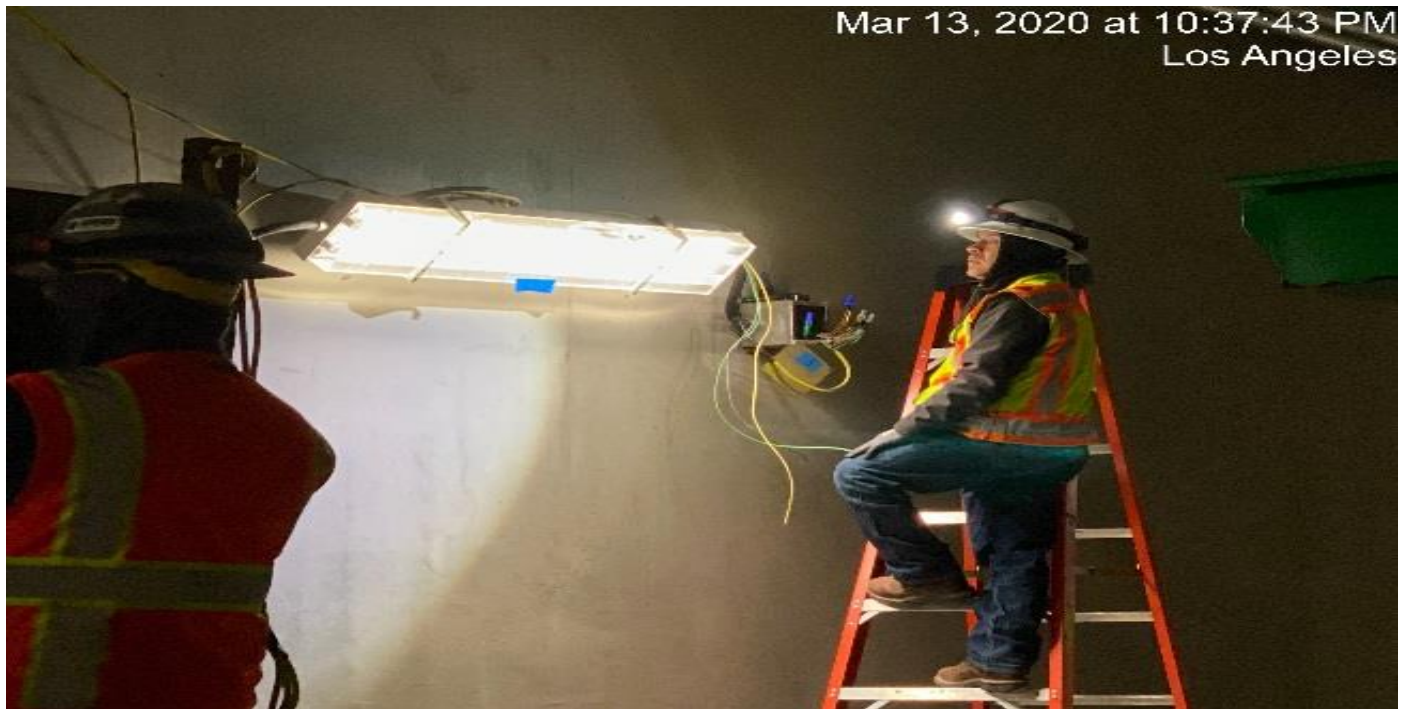
UG-4- – Continue pulling wire for the emergency lighting along the northbound tunnel at Sta 379+00.
