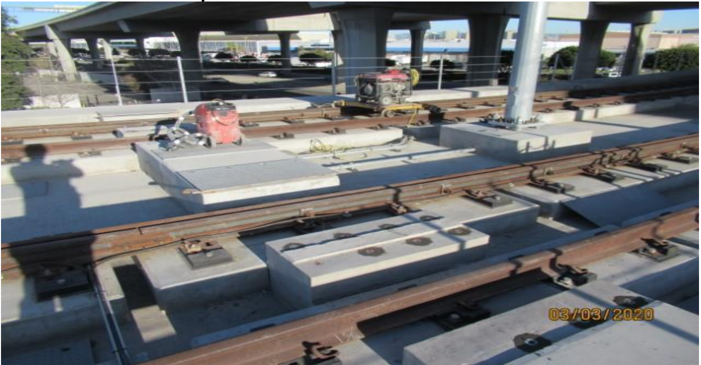
GUIDEWAY - WSCC setting up workstation for grinding insert epoxy on inserts for crossing on west leg of wye STA 13+01.
