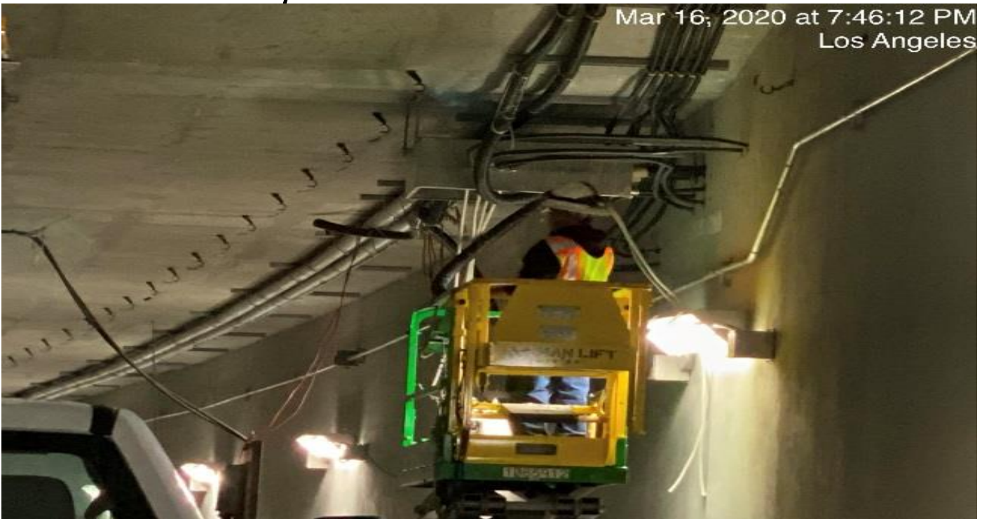
UG-4- Continue pulling wire for the emergency lighting along the southbound tunnel.
