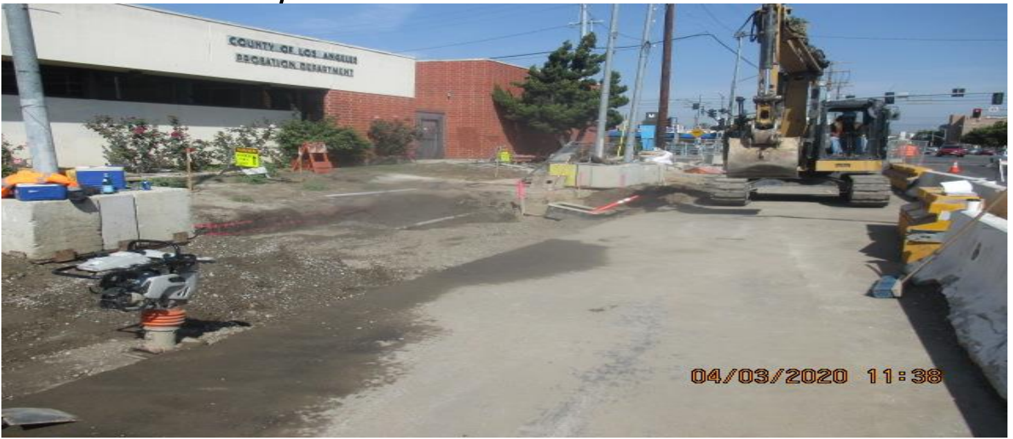
EXPO STATION- Excavating for new curb/gutter and sidewalk installation on Crenshaw Blvd between Exposition Blvd and Rodeo Blvd. 3/4/20
