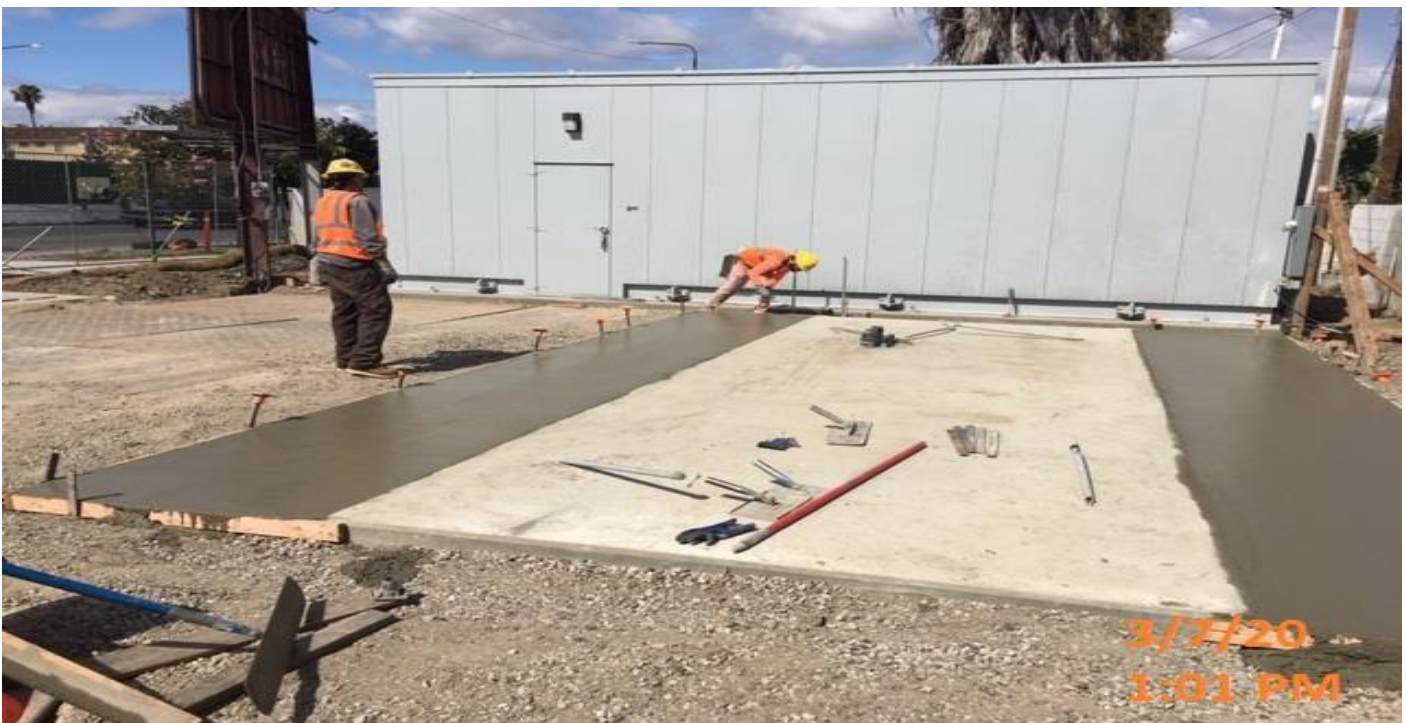
Park Mesa – Continued placing concrete for the generator pads at TPSS#7 on 60th St & Crenshaw Blvd.
