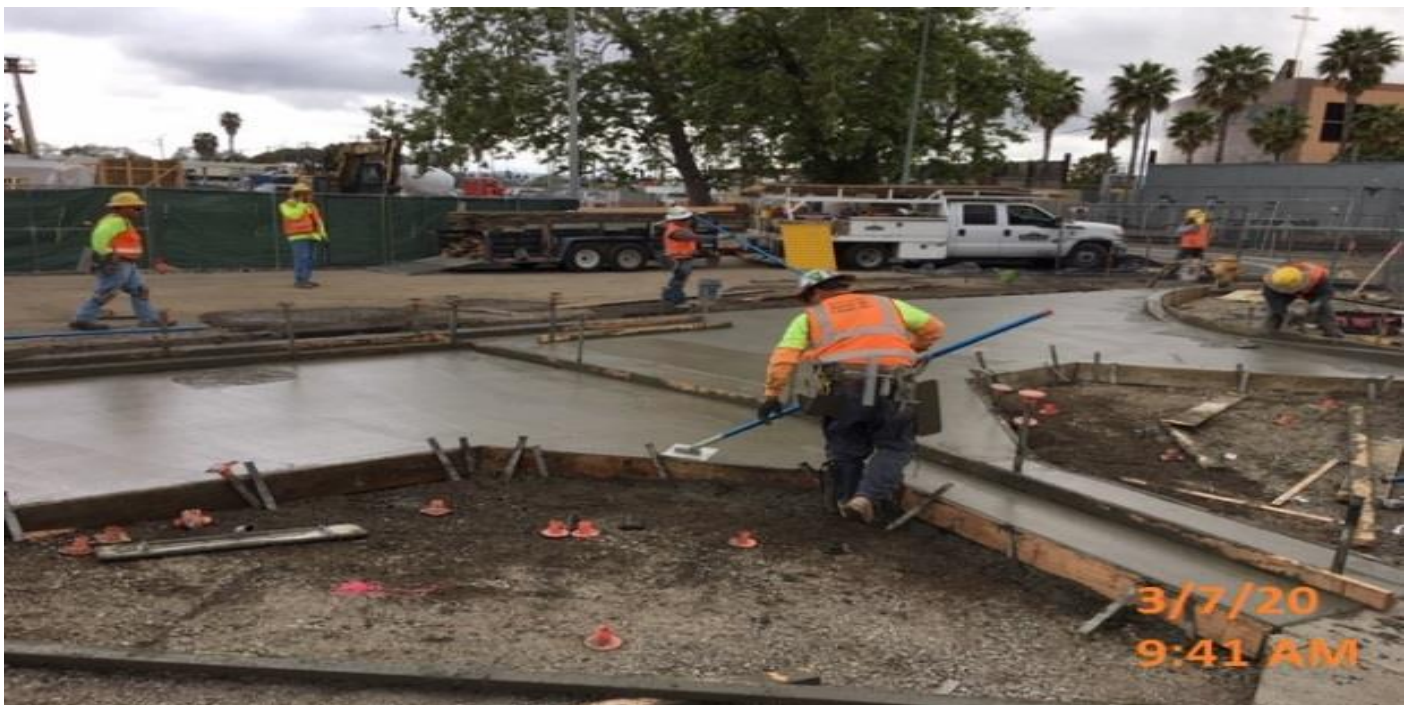
EXPO STATION- Placing concrete for cross gutter on Bronson St. east of the plaza.
