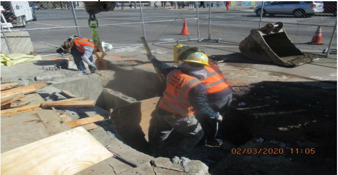
EXPO STATION- Began roof deck formwork for Catch Basin #19 on the northeast corner of Exposition Blvd and Crenshaw Blvd. 3/2/20
