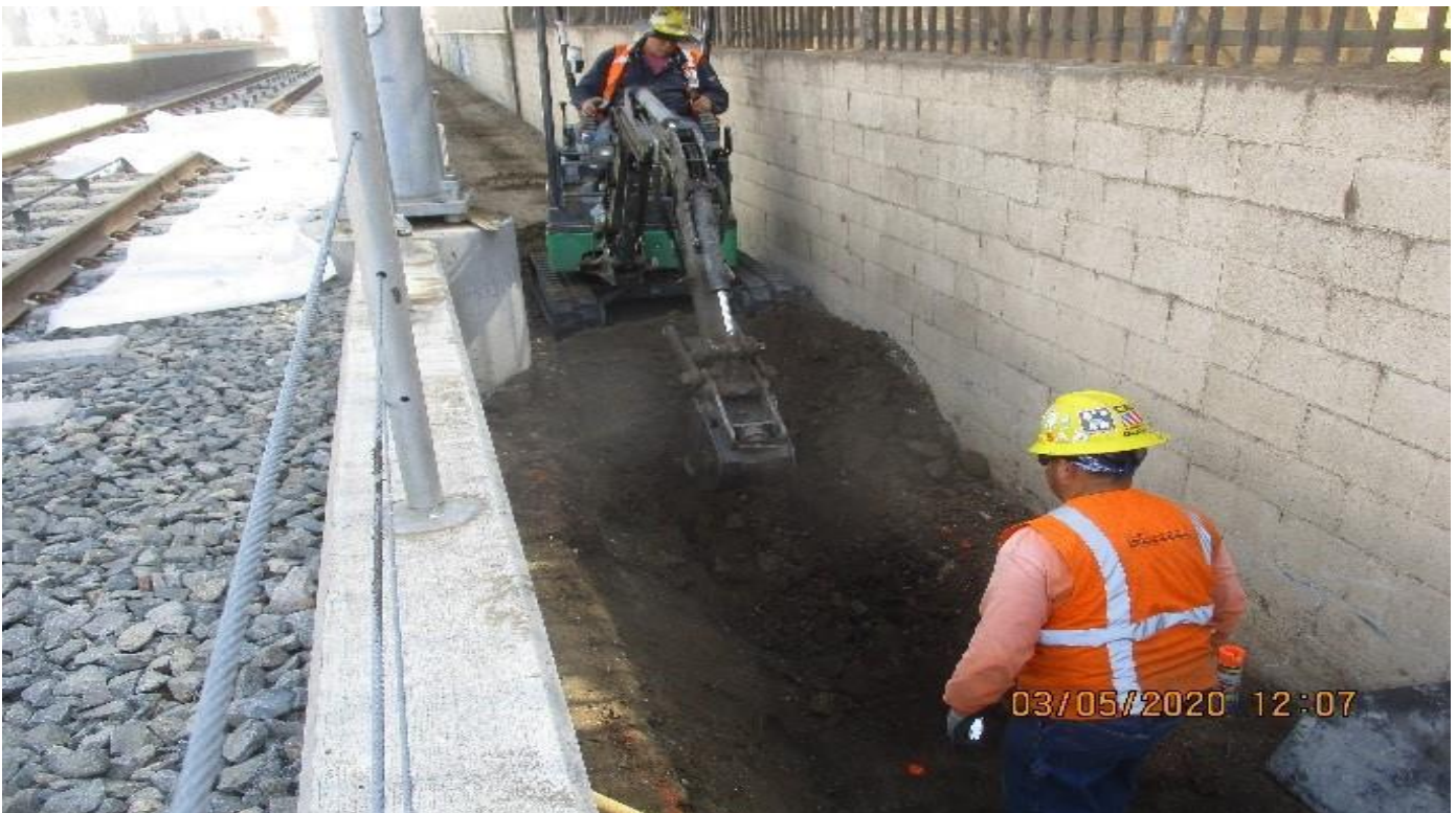
WEST Blvd - Soil backfilled Continued digging V ditch behind ballast wall at West Station.
