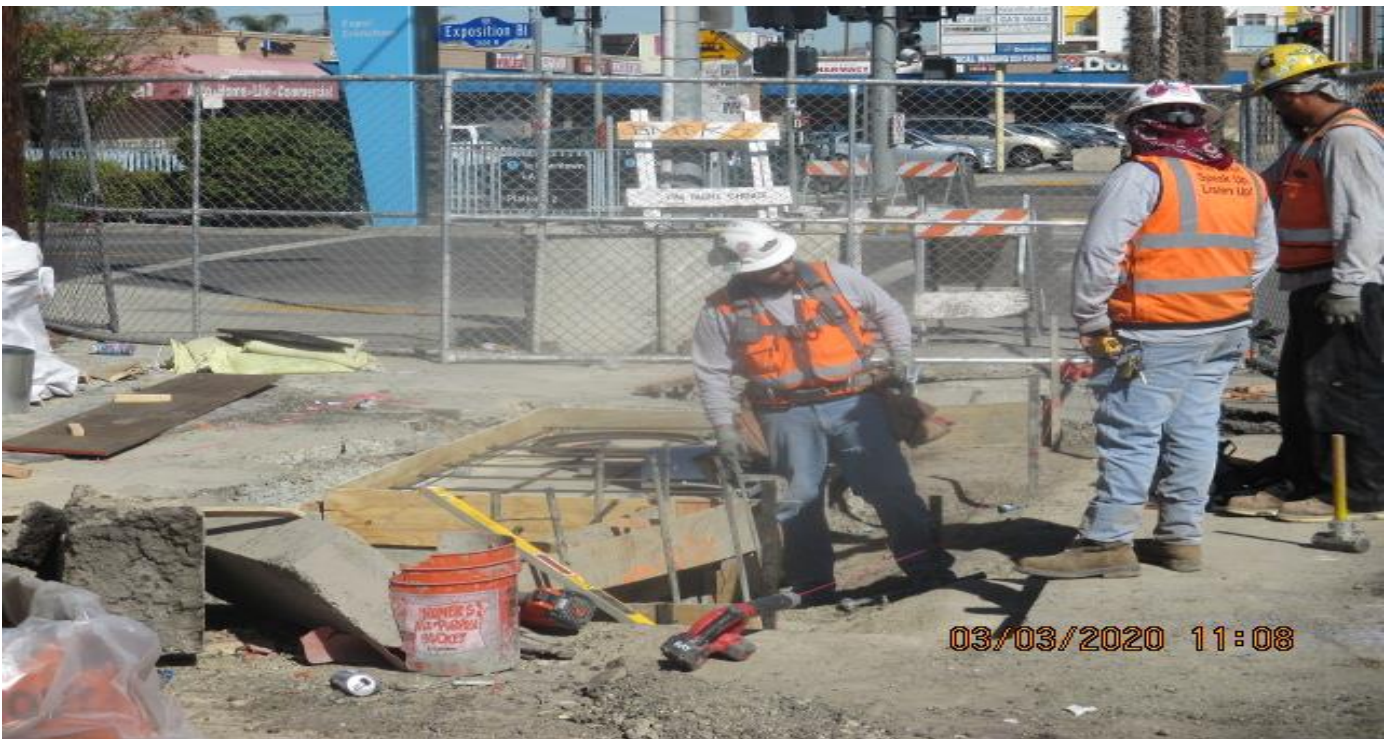
EXPO STATION- Continue roof deck formwork for Catch Basin #19 on the northeast corner of Exposition Blvd and Crenshaw Blvd. 3/3/20
