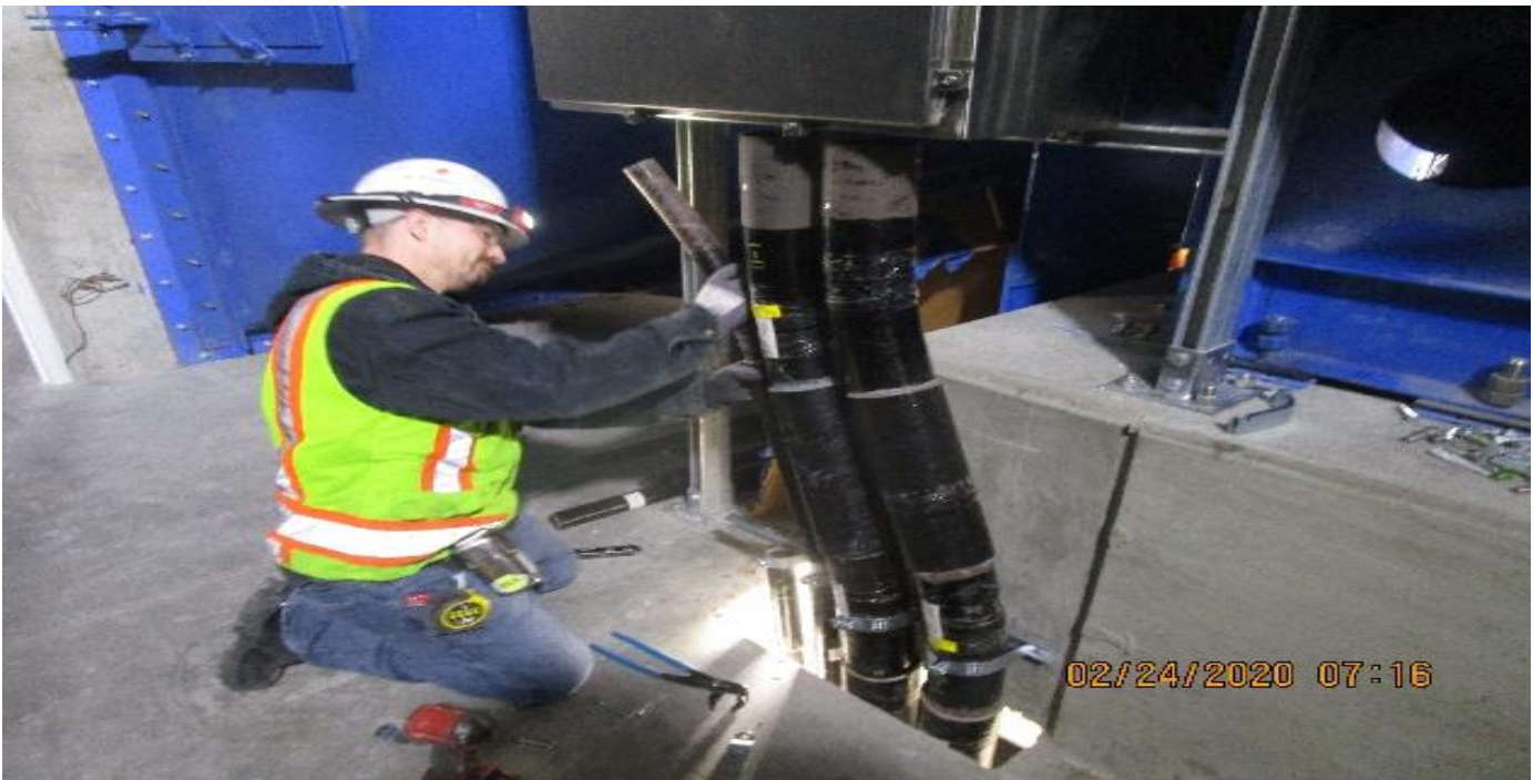
LEIMERT PARK STATION – Installing conduit to the pull box for EVF-6-101 in the South Fan Room C – 102 of the concourse level.
