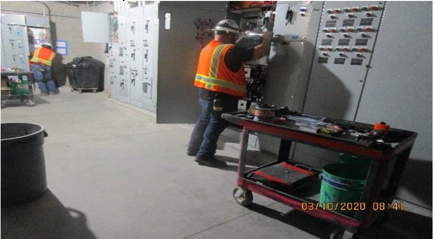
MLK STATION - MLK, Aux power (S) C109, Continued at MCC1,S & MCC2,S pre-energization Q,C check list items.
