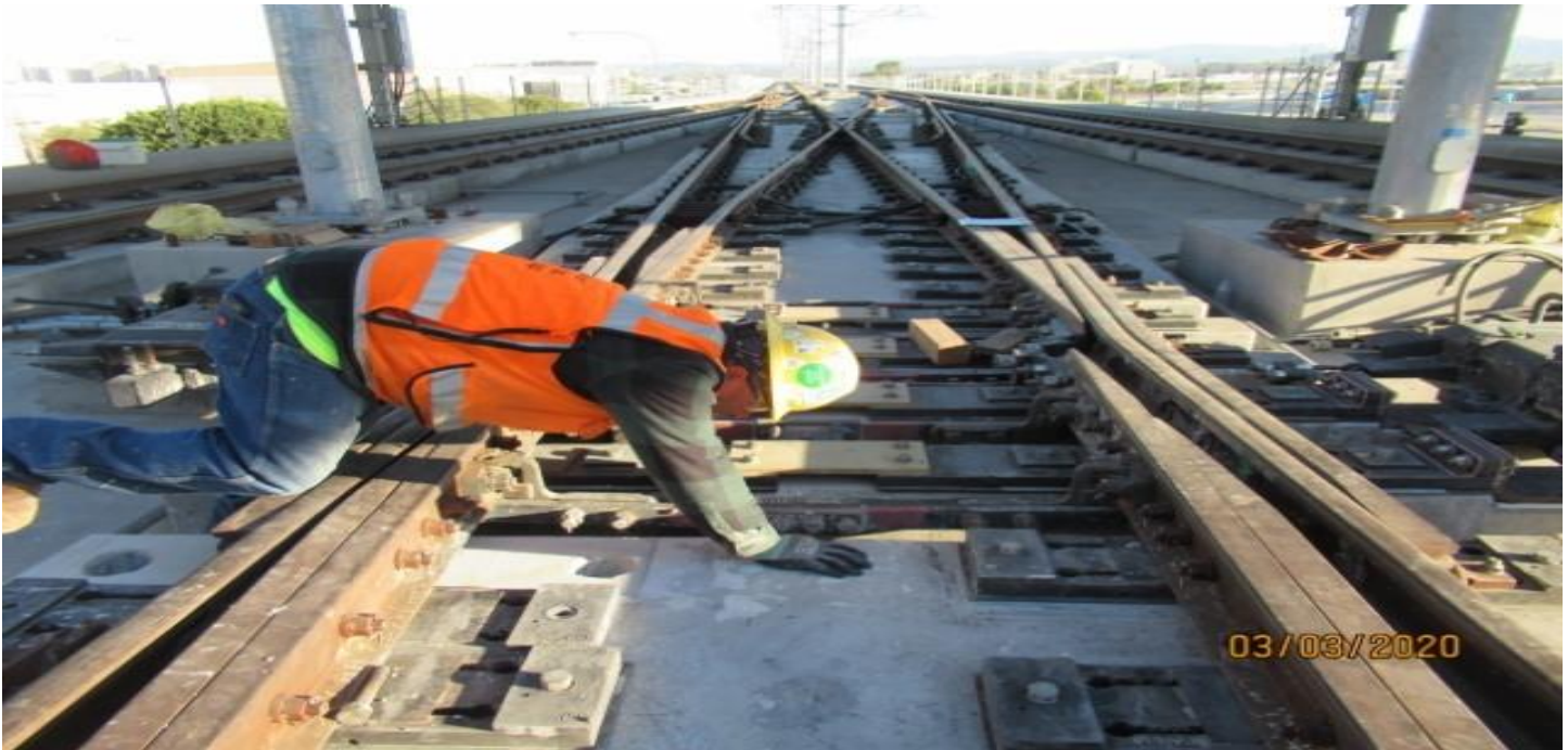
GUIDEWAY - WSCC Concrete foreman checking elevation differences between gauge & field side of slab on MPF at GL Wye STA 13+90
