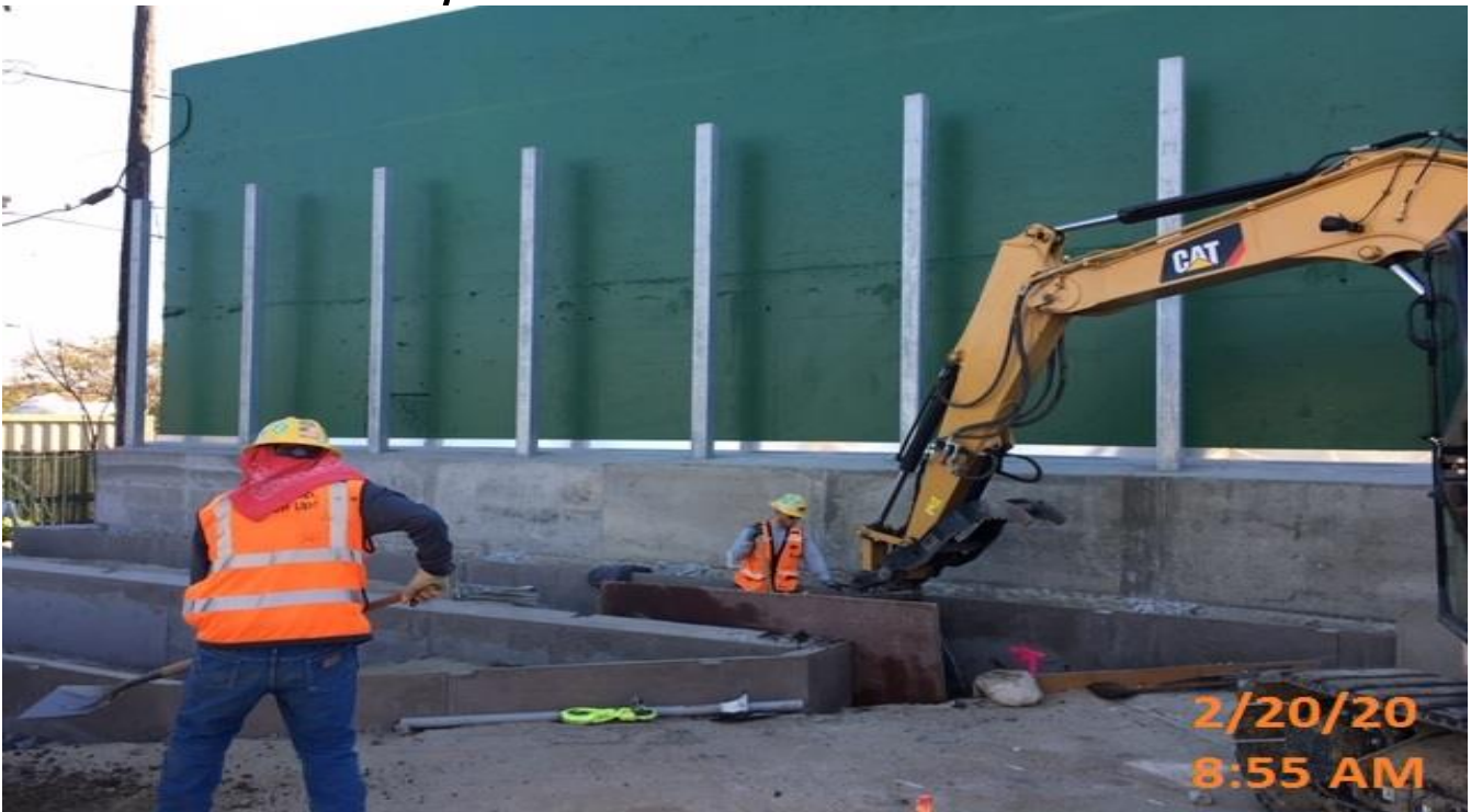
LEIMERT PARK STATION – Excavating for ADA ramp installation at the southeast end of the plaza level.
