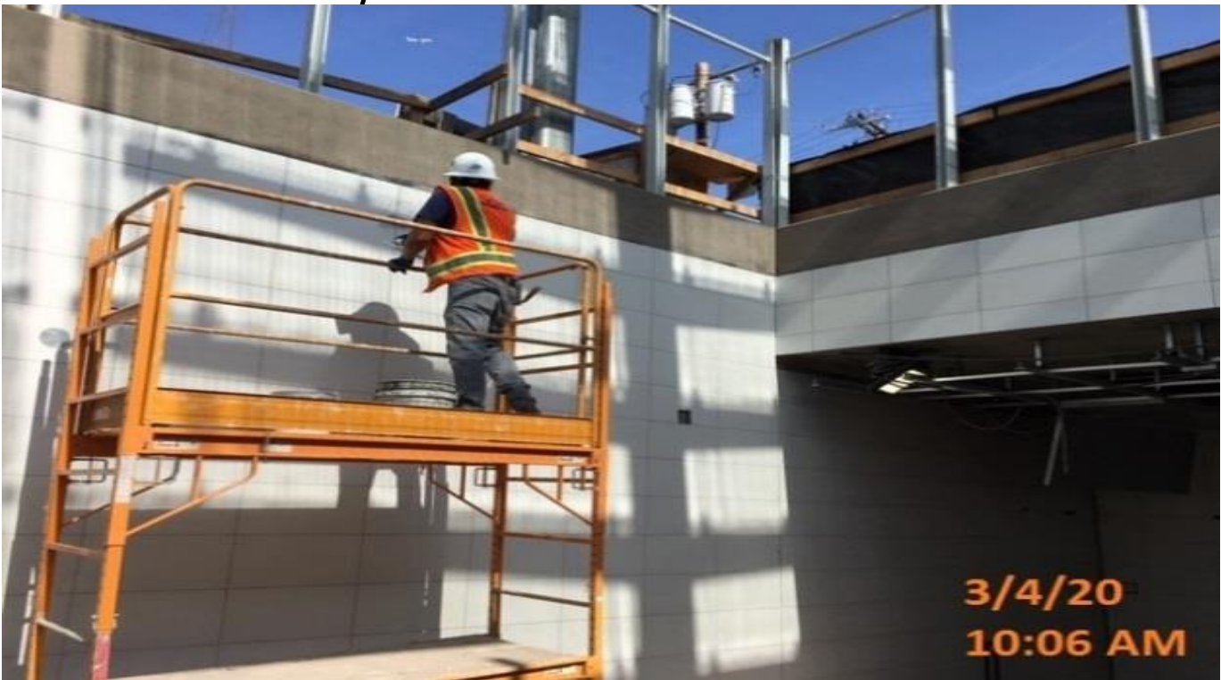
LEIMERT PARK STATION – Resume installation of remaining miscellaneous wall tiles at the plaza level.
