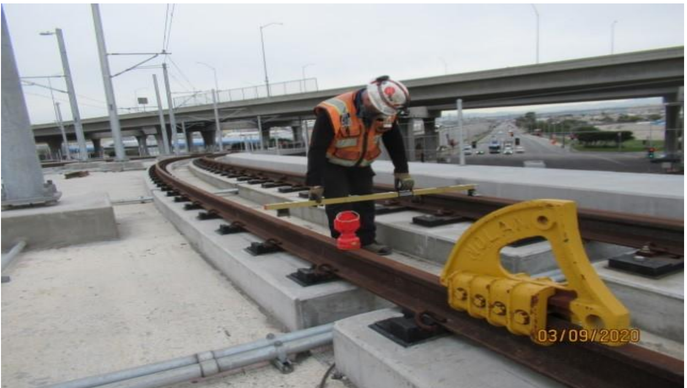
GUIDEWAY - WSCC QC track inspector verifying cross level & track gauge on NB1300 track GL Wye STA 10+75 .
