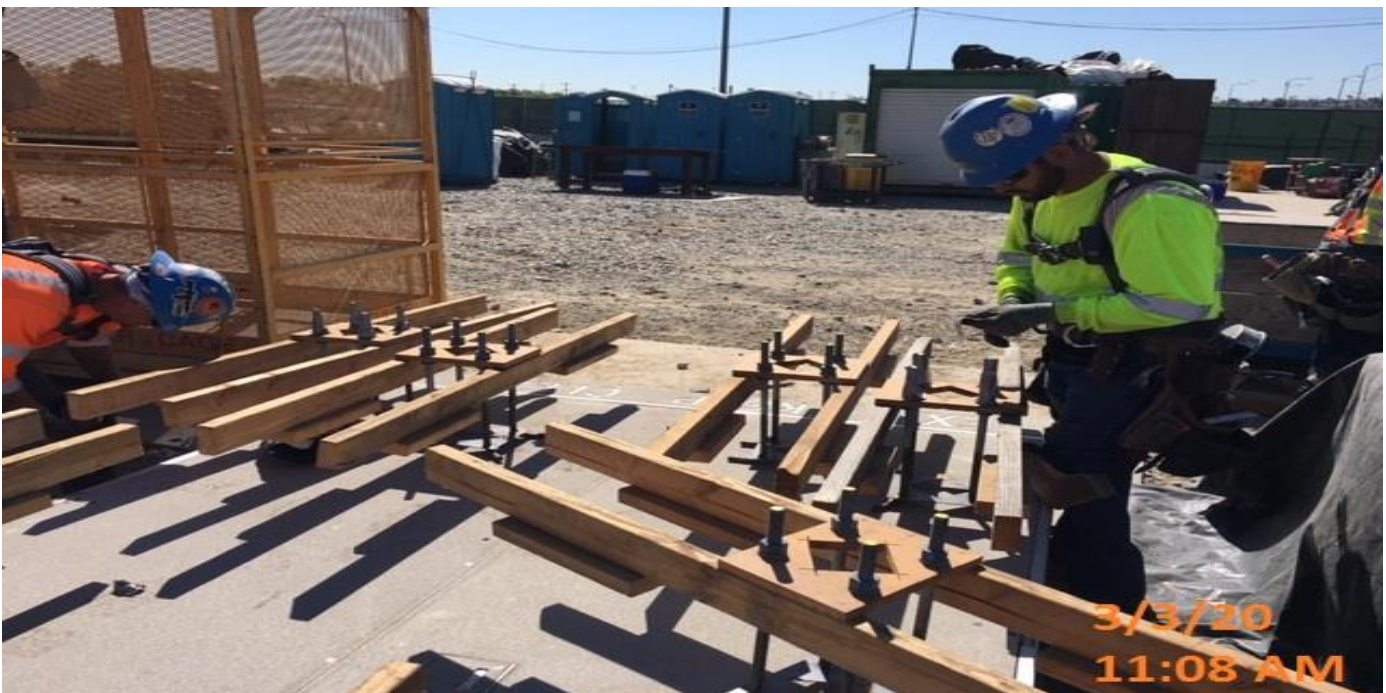
EXPO STATION – Continued setting sonotube foundation forms and bolt template for the installation of the luminaire light posts at the plaza level.
