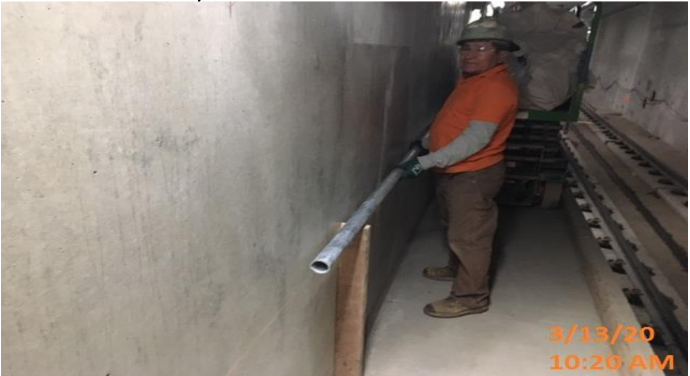
UG3 – Installing handrails for the emergency walkway on the southbound tunnel at Sta 287+50.
