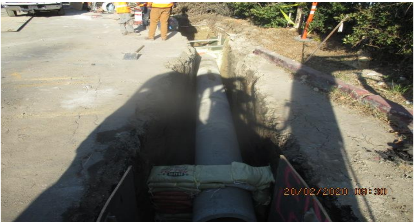
EXPO STATION – Continue installing sections of 18” RCP for Line B – storm drain at the Cul-de-sac on Bronson St. east of the plaza. 2/20/20
