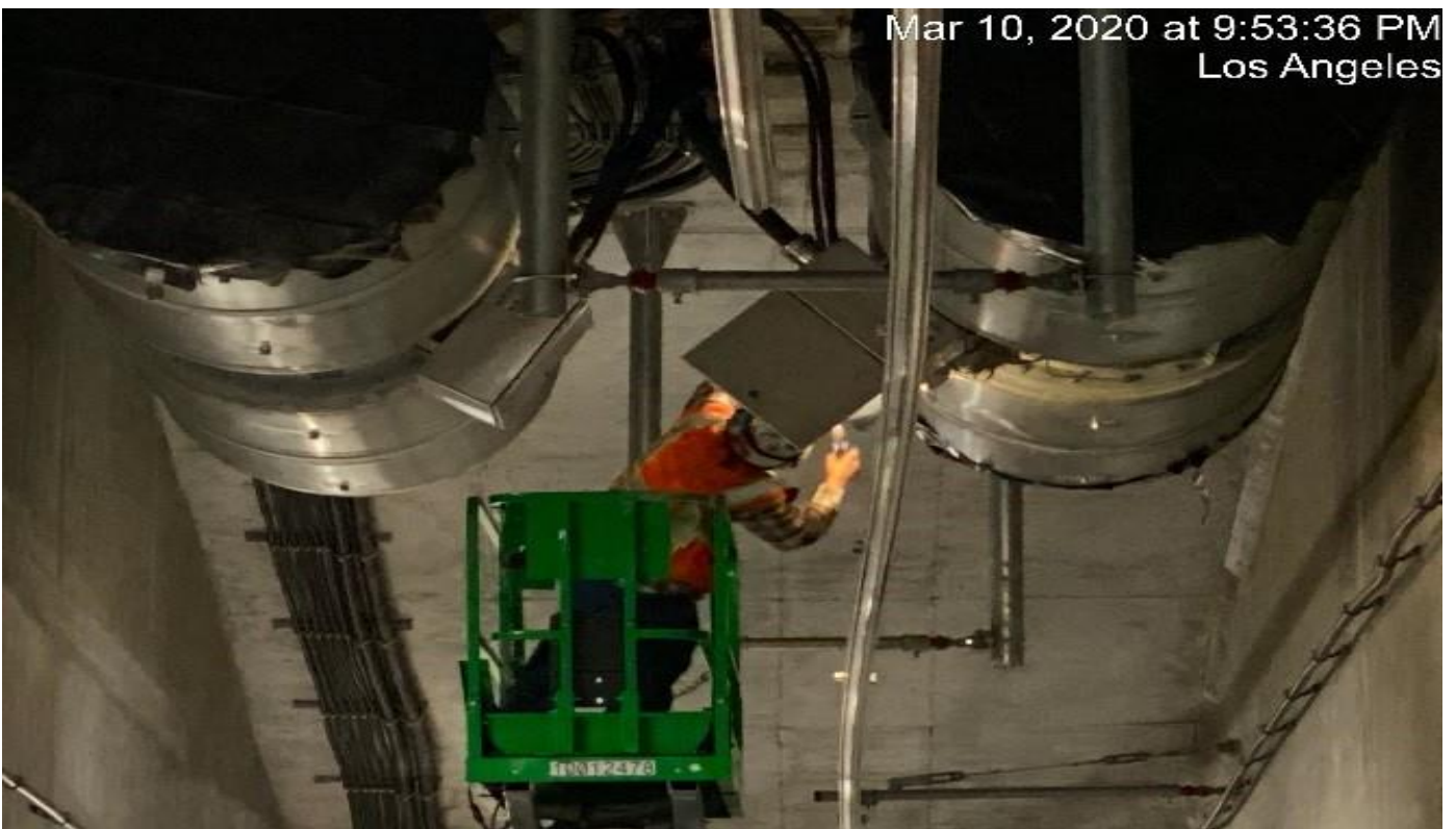
UG3 – DCD connecting wires for Booster fans northbound UG-3
