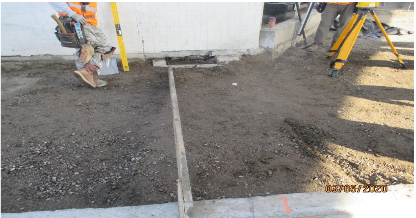
MANCHESTER AVE- Parking lot drain that was forgotten on Manchester. Facing north.
