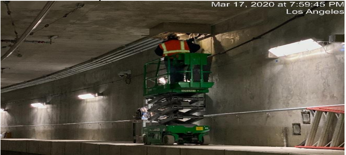
UG3 – Continue splicing wires for the tunnel booster junction boxes at the southbound tunnel at Sta 283+30.
