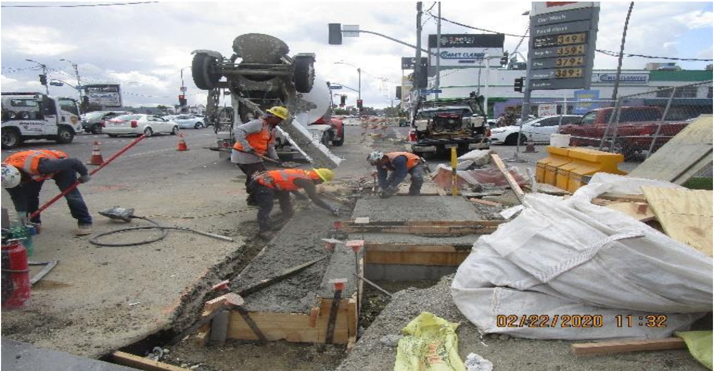
EXPO STATION- Placing concrete for Catch Basin #16 on the southbound side of Rodeo Blvd and Crenshaw Blvd.
