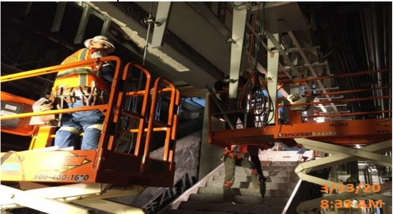
MLK STATION - Continue installing steel stud track and framing underneath escalator 3&4 at the platform level.
