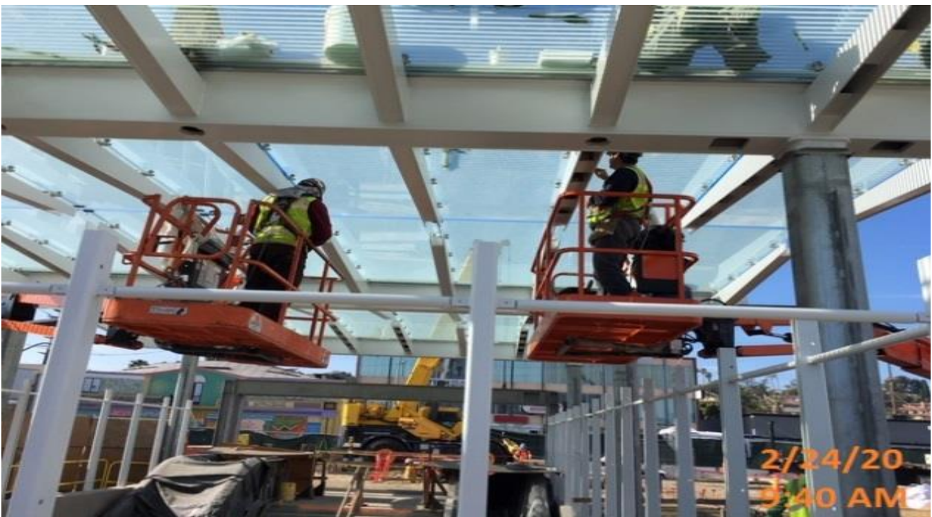
LEIMERT PARK STATION – Continue glass panel installation and sealing edges with silicone above the main entrance canopy structure at the plaza level.
