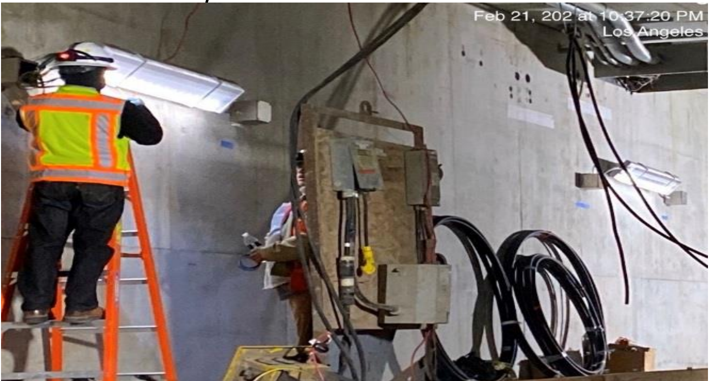
UG4 – Continue pulling wire for the emergency lighting along the northbound tunnel at Sta 376+50.
