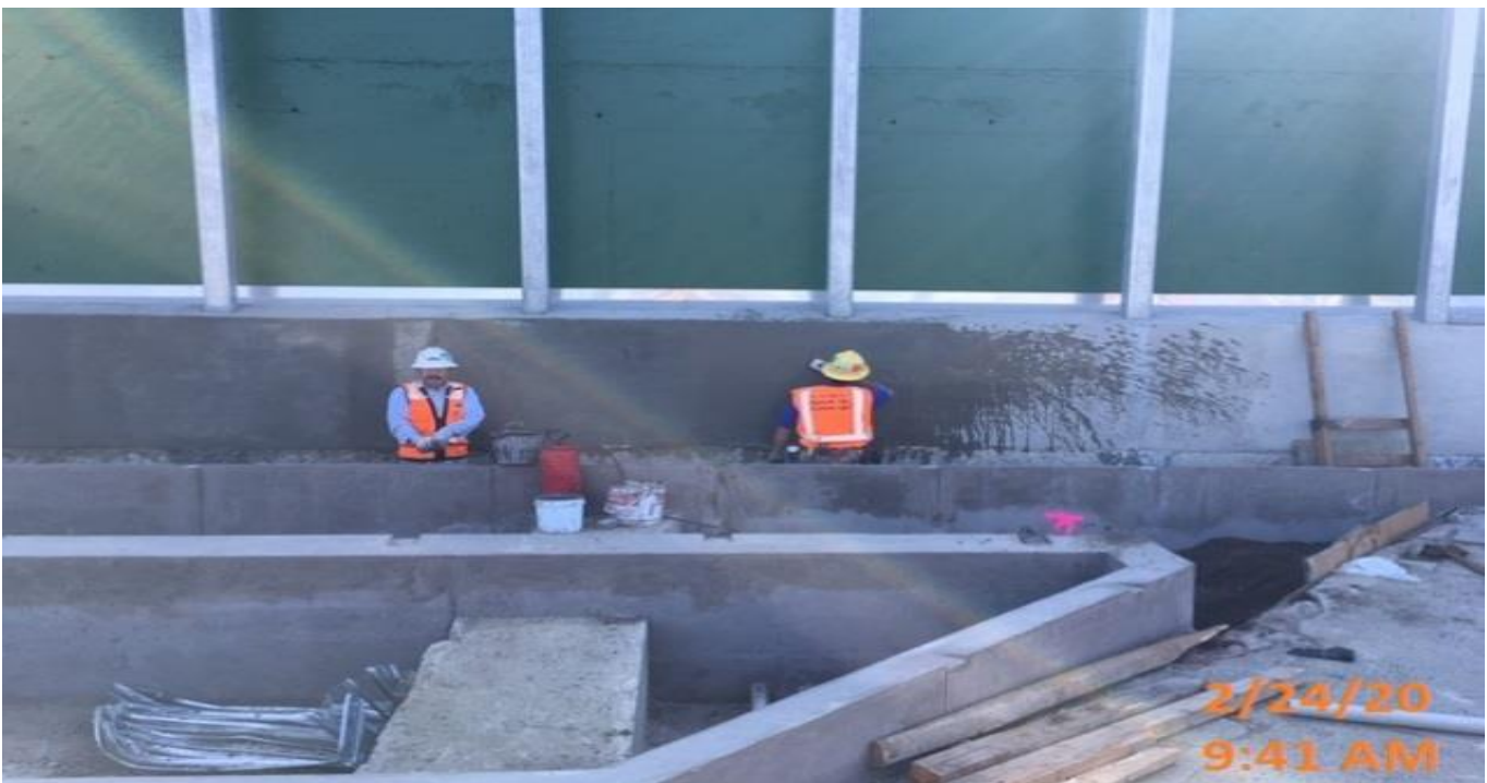
LEIMERT PARK STATION – Surfacing and patching the green screen wall at the south perimeter of the plaza level.
