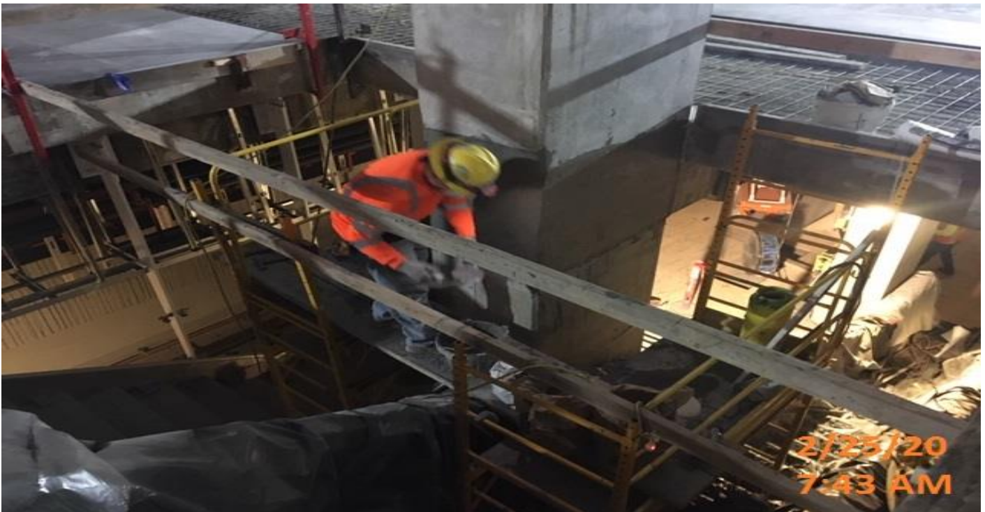
MLK STATION – Surfacing and patching the architectural columns at the concourse level.
