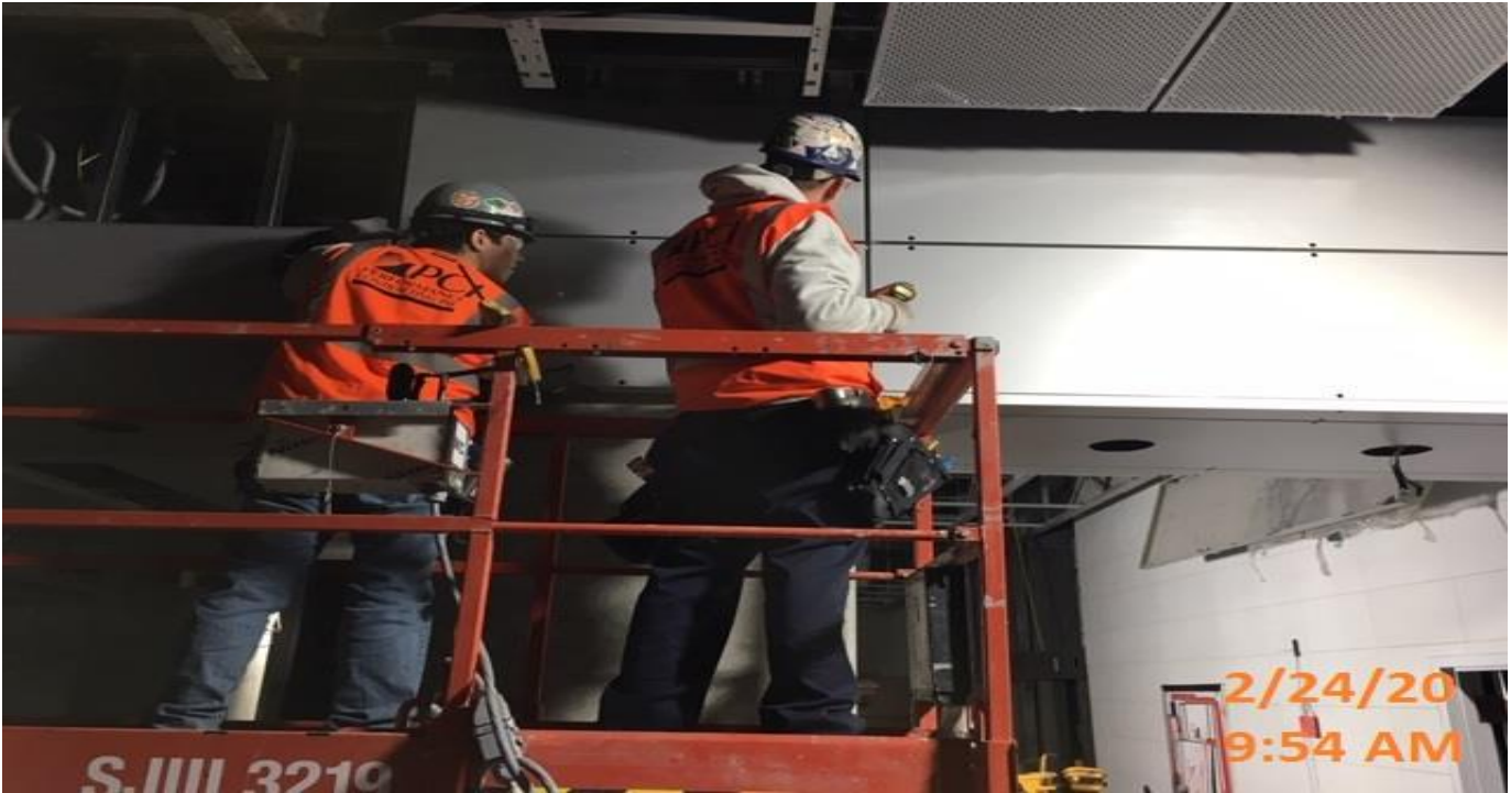
LEIMERT PARK STATION – Installing aluminum ceiling panels throughout the Free & Paid Area of the concourse level.
