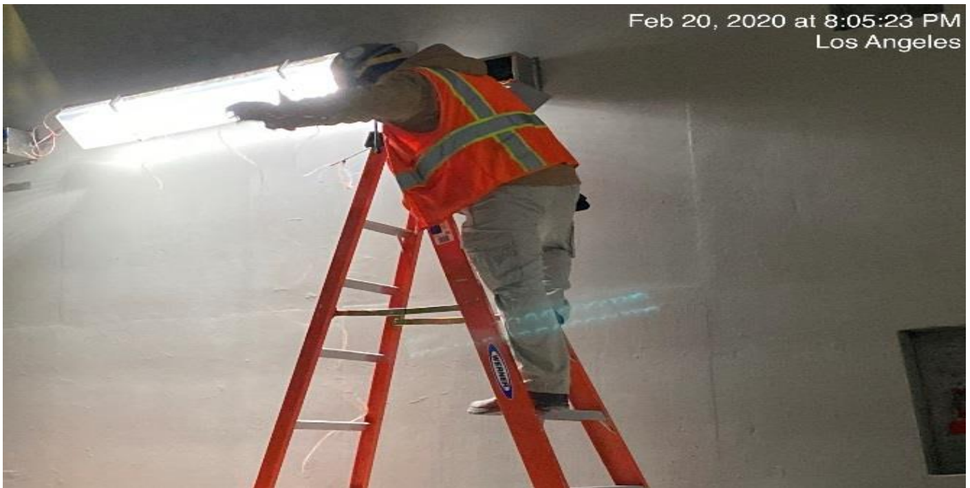
UG4 – Continue pulling wire for the emergency lighting along the northbound tunnel at Sta 374+85.
