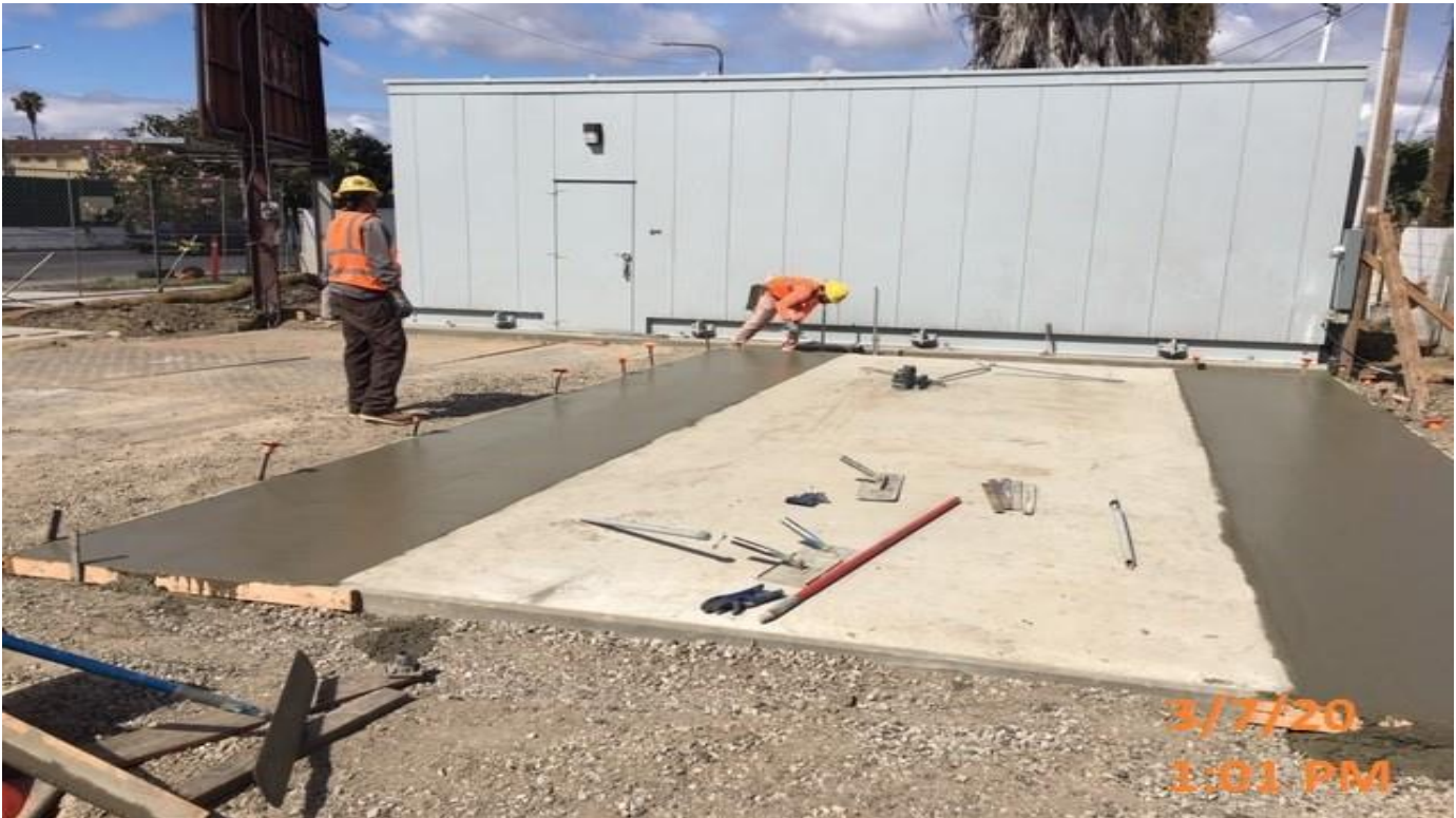
UG3 – UG3. Aux. Site – WSCC crew placing concrete for generator pad walkway
