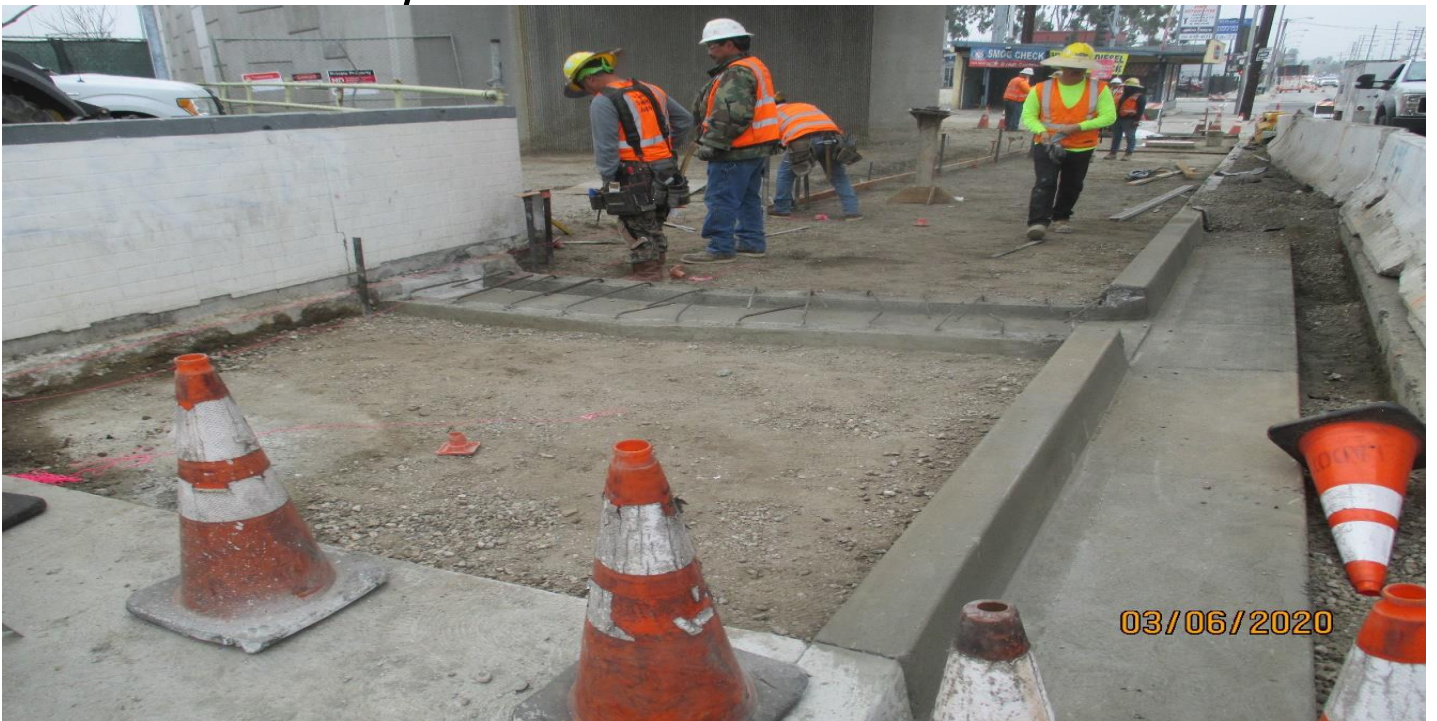
MANCHESTER AVE- Parking lot drain in the sidewalk on the north side of Manchester.
