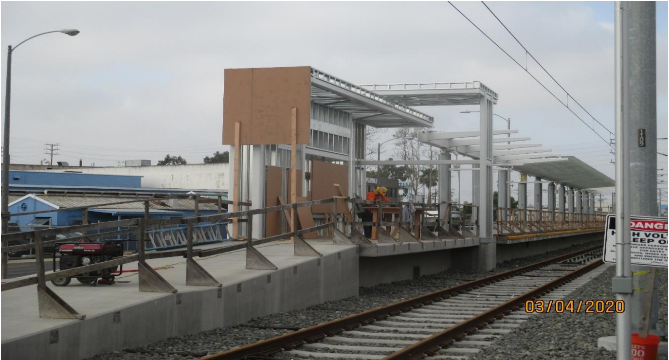
HINDRY AVE- Ticket vending machine mock-up construction at the Hindry Station NB platform.
