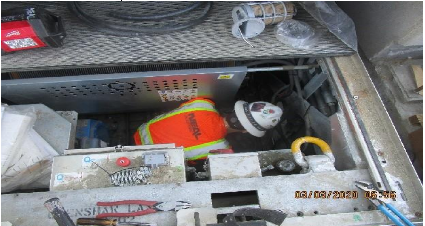
Crenshaw/Vernon – Vernon, Concourse, Escalator 3 & 4 lower pits, begin rough in JB's, GRC & seal tight service light, switch & receptacles.
