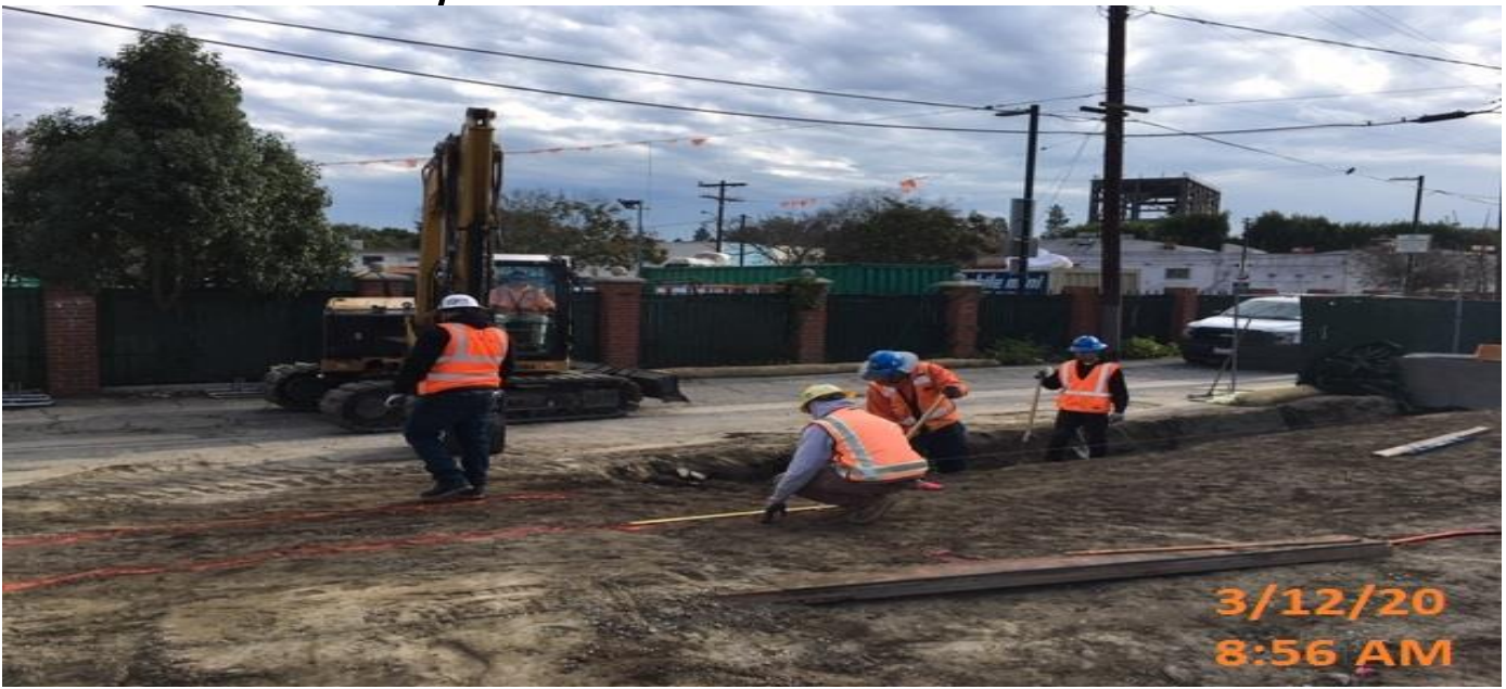
LEIMERT PARK STATION – Continue excavating for the east emergency exit staircase and planter wall section at the plaza level.
