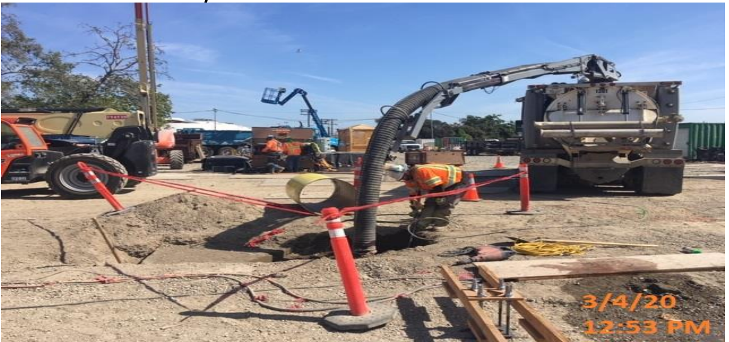
EXPO STATION- Continue setting sonotube foundation for the installation of the luminaire light posts at the plaza level.
