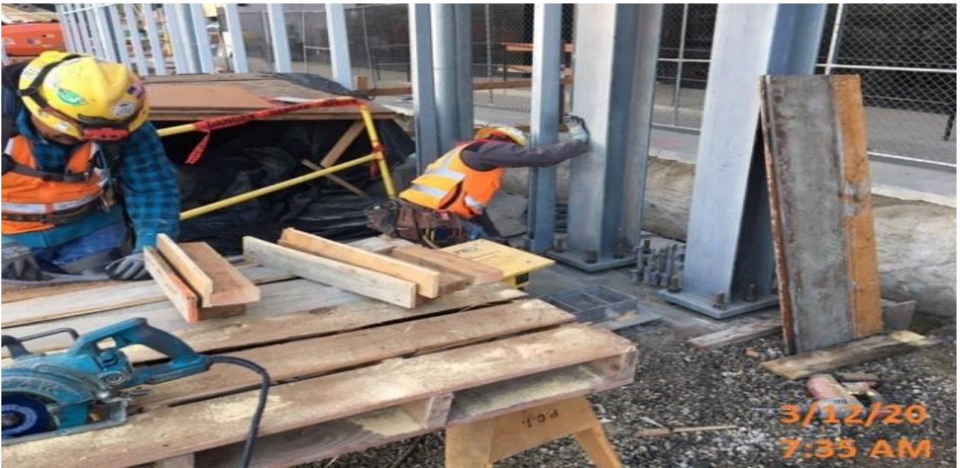
MLK STATION - Building forms for metal base plates for the main entrance canopy columns at the plaza level.
