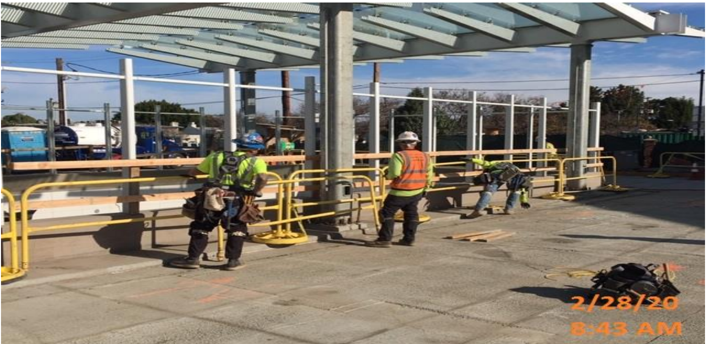
LEIMERT PARK STATION – Began perimeter formwork for slab encasement of irrigation lines for the main entrance canopy at the plaza level.
