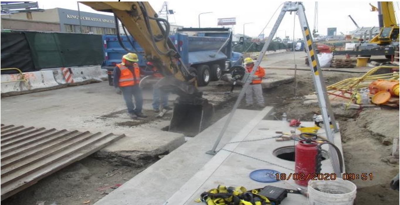
MLK STATION – Continue sack/patch and ladder installation of Catch Basin #3 at the northeast corner of the plaza level. 2/18/20
