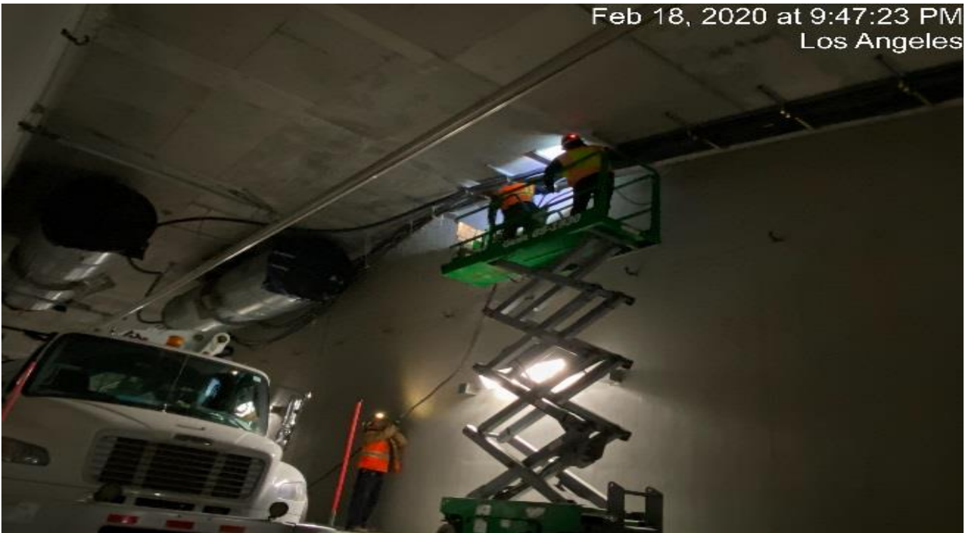
UG4 – Continue wiring and running cable for the booster fans in the northbound tunnel at Sta 374+25.
