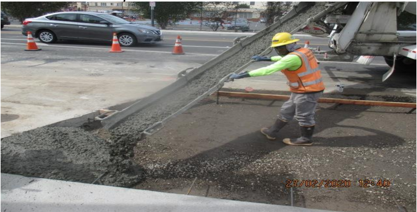
Park Mesa – Placing concrete for the bus pad installation on the southeast corner of 60th St & Crenshaw Blvd. 2/27/20
