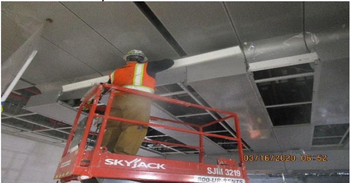
LEIMERT PARK STATION – Continued installing light cove and ceiling panels throughout the Free & Paid Area of the concourse level.
