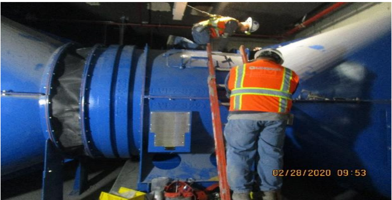
MLK STATION – Began flex connection installation for EVF-6-322 in the North Fan Room C – 142 of the concourse level.
