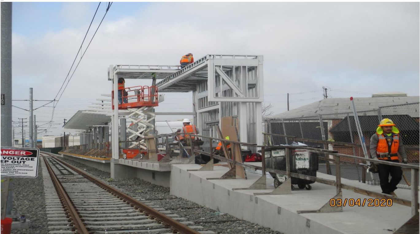
HINDRY AVE- Ticket vending machine mock-up construction and metal stud framing at the Hindry Station SB platform.
