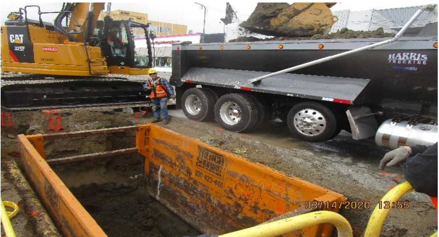
EXPO STATION- Excavated and completed the installation of shoring box #1 for the oil water separator on Rodeo Blvd and Crenshaw Blvd.
