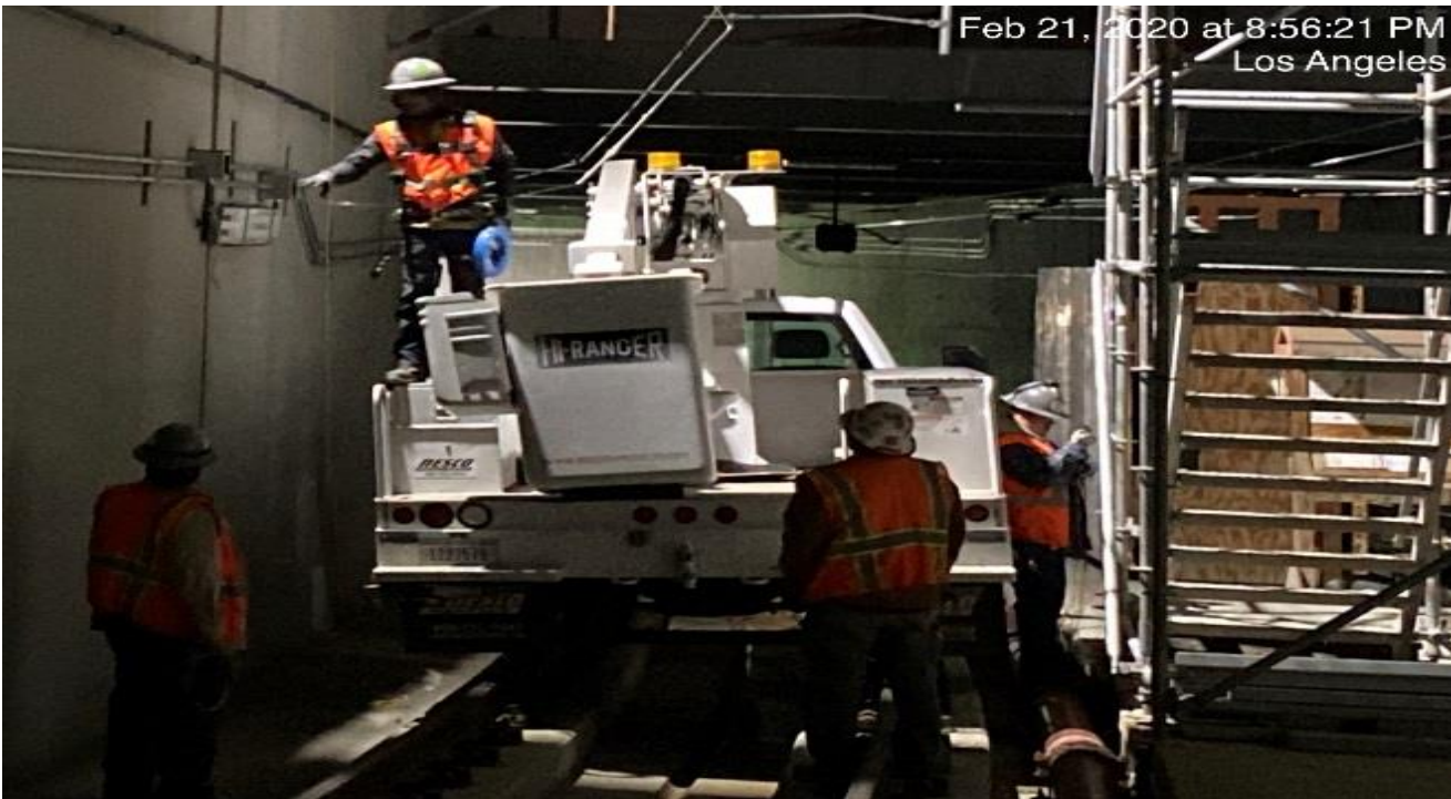
UG3 – Continue pulling wire for the emergency lighting at the south end portal entrance.
