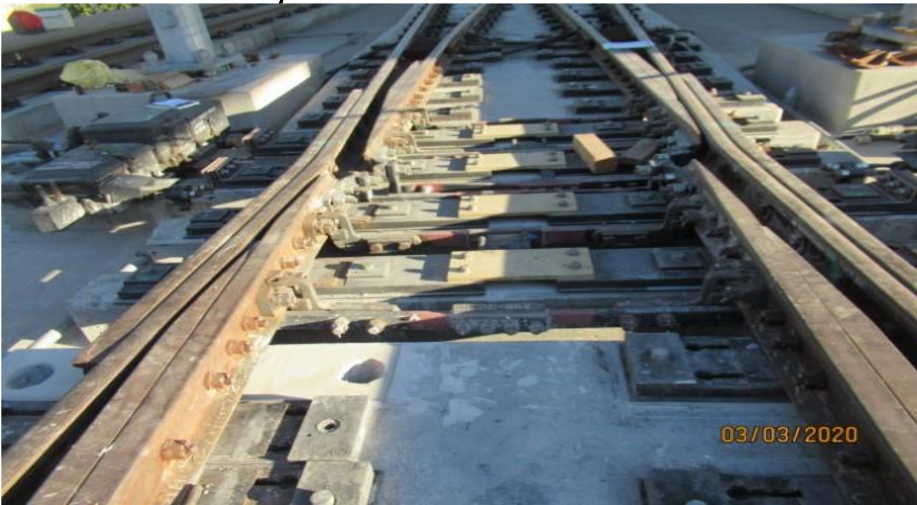
GUIDEWAY - MPF at GL Wye STA 13+90 incomplete work on concrete.
