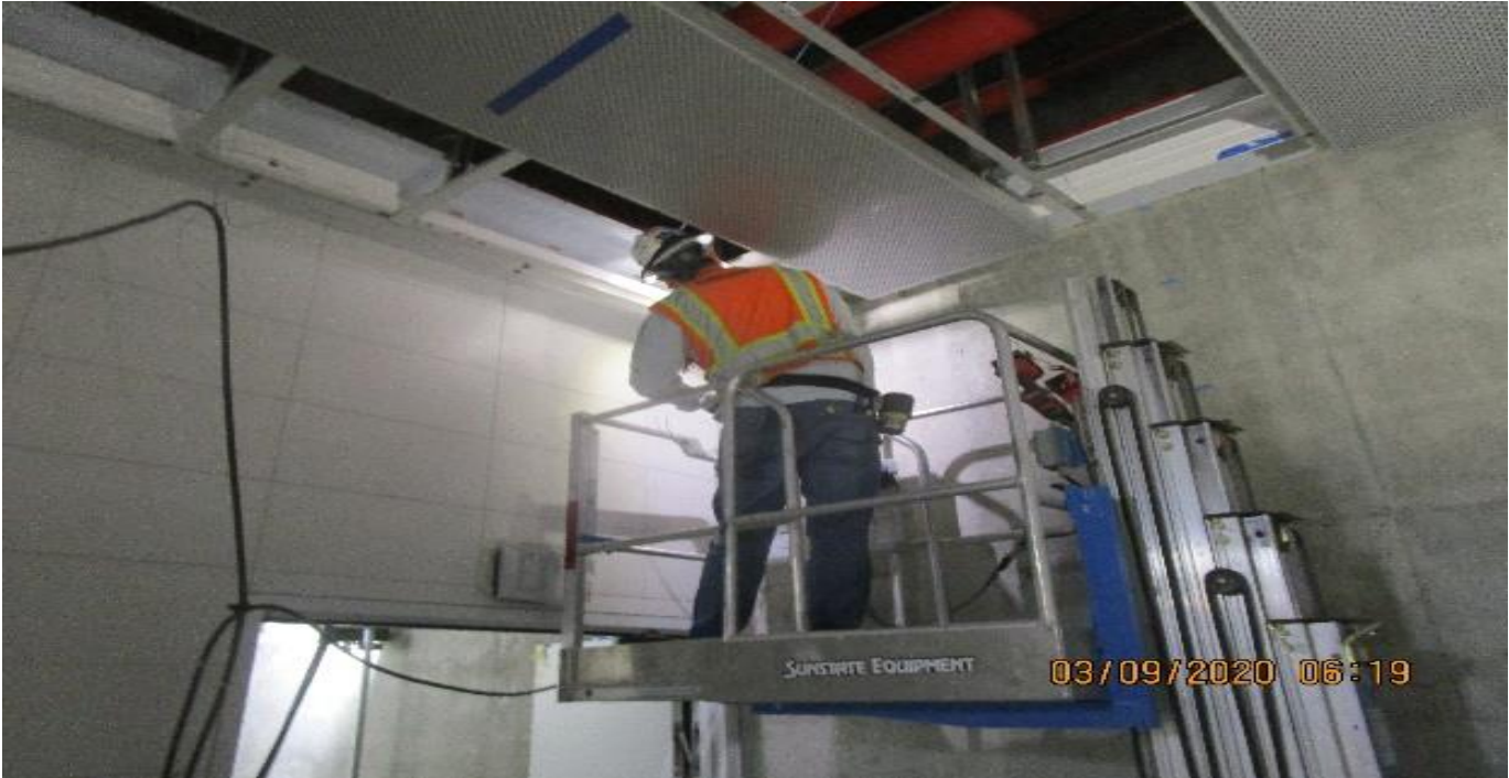
LEIMERT PARK STATION – Continued installing light cove and ceiling panels throughout the Free & Paid Area of the concourse level.
