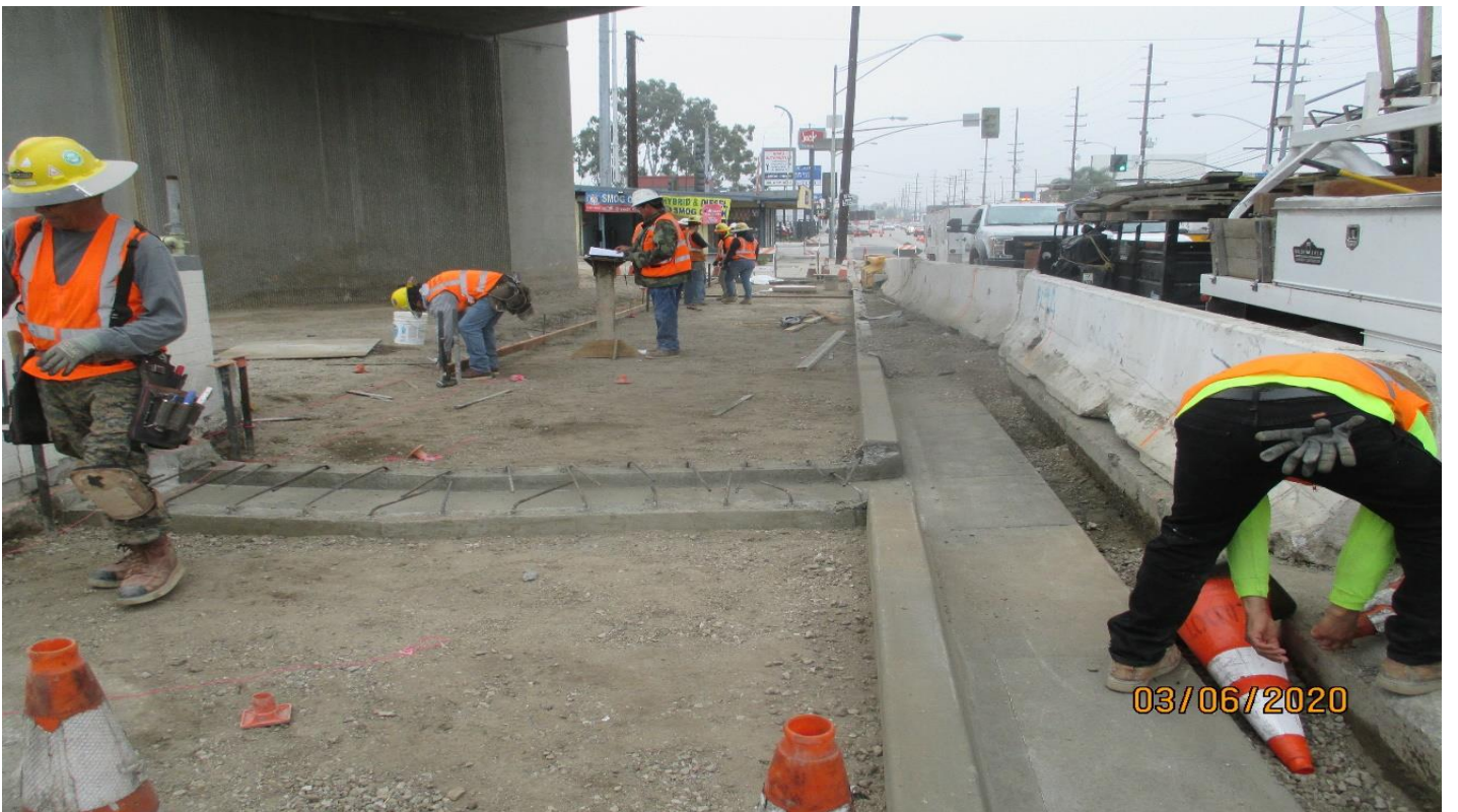
MANCHESTER AVE- Forming for concrete for the sidewalk on the north side of Manchester.
