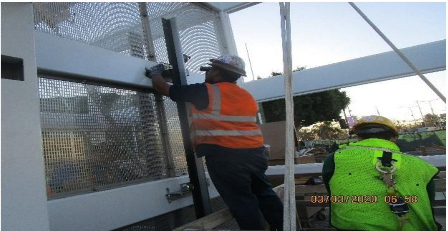
Crenshaw/Vernon – Vernon, Elevator hoist way #1, Continued install guide rail brackets, plumb, square & align top out guide rails.
