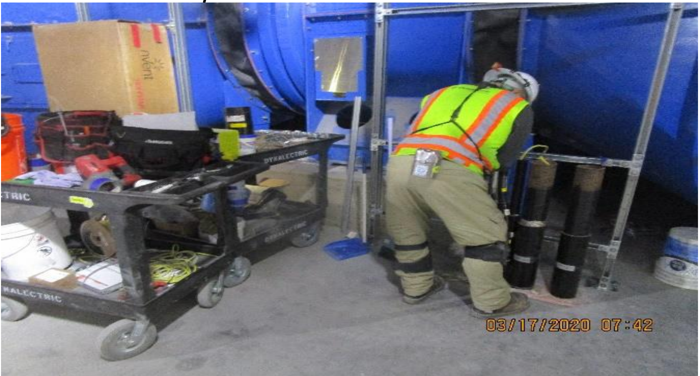
MLK STATION - Continue rough in for fire rated conduit installation to the pull box for EVF-7-121 in the South Fan Room C – 102 of the concourse level.
