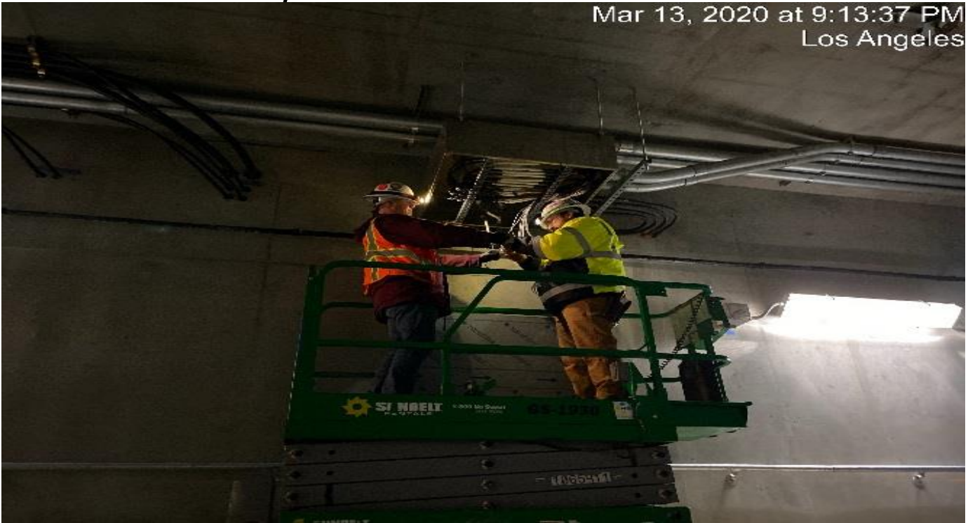
UG3 – Continue splicing wires for the tunnel booster junction boxes at the southbound tunnel at Sta 286+30.
