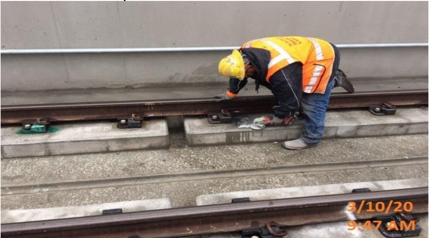
UG3 – UG3 – WSCC crew grinding numbers off of plinths along SB side.
