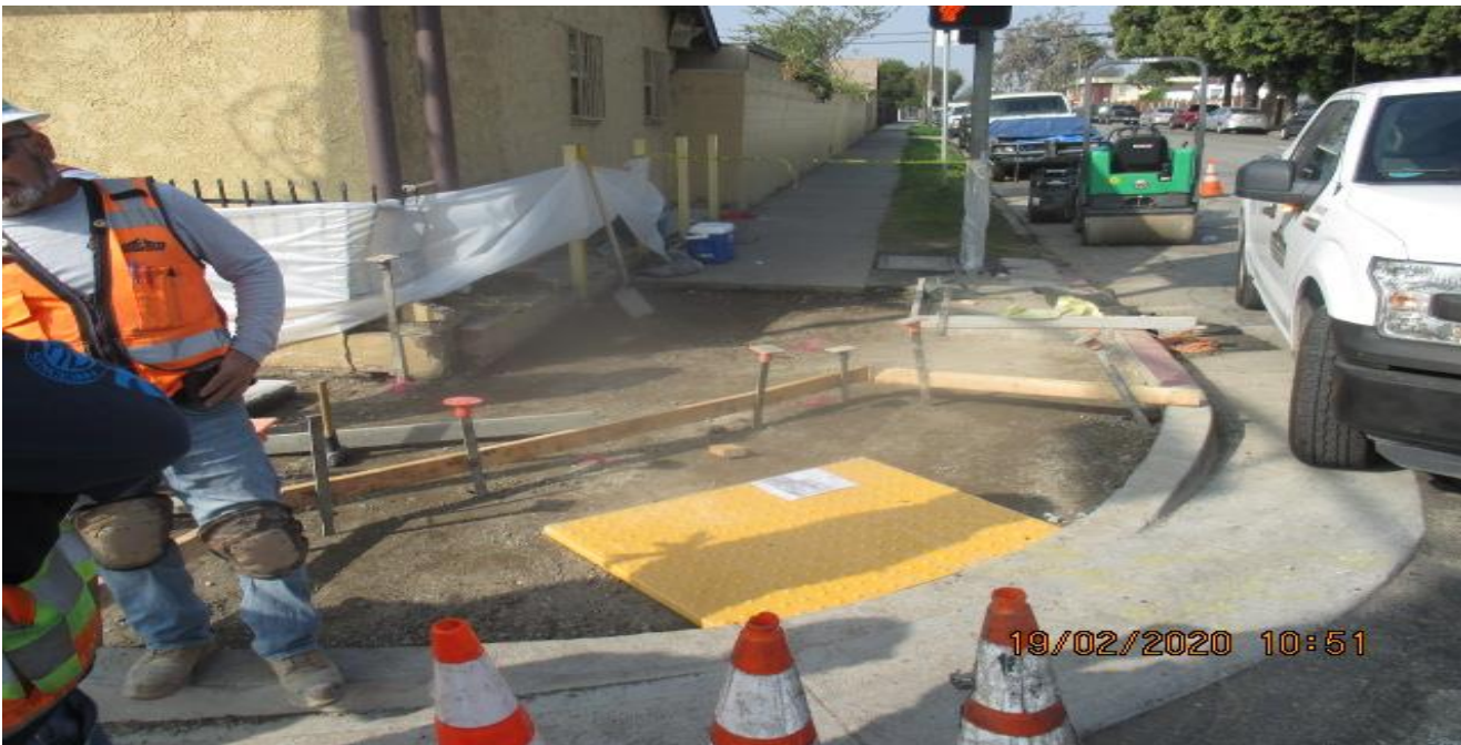
Park Mesa – Installing block-out forms in preparation for new concrete placement of sidewalk and ADA ramp on the southwest corner 63rd St and Crenshaw Blvd. 2/19/20
