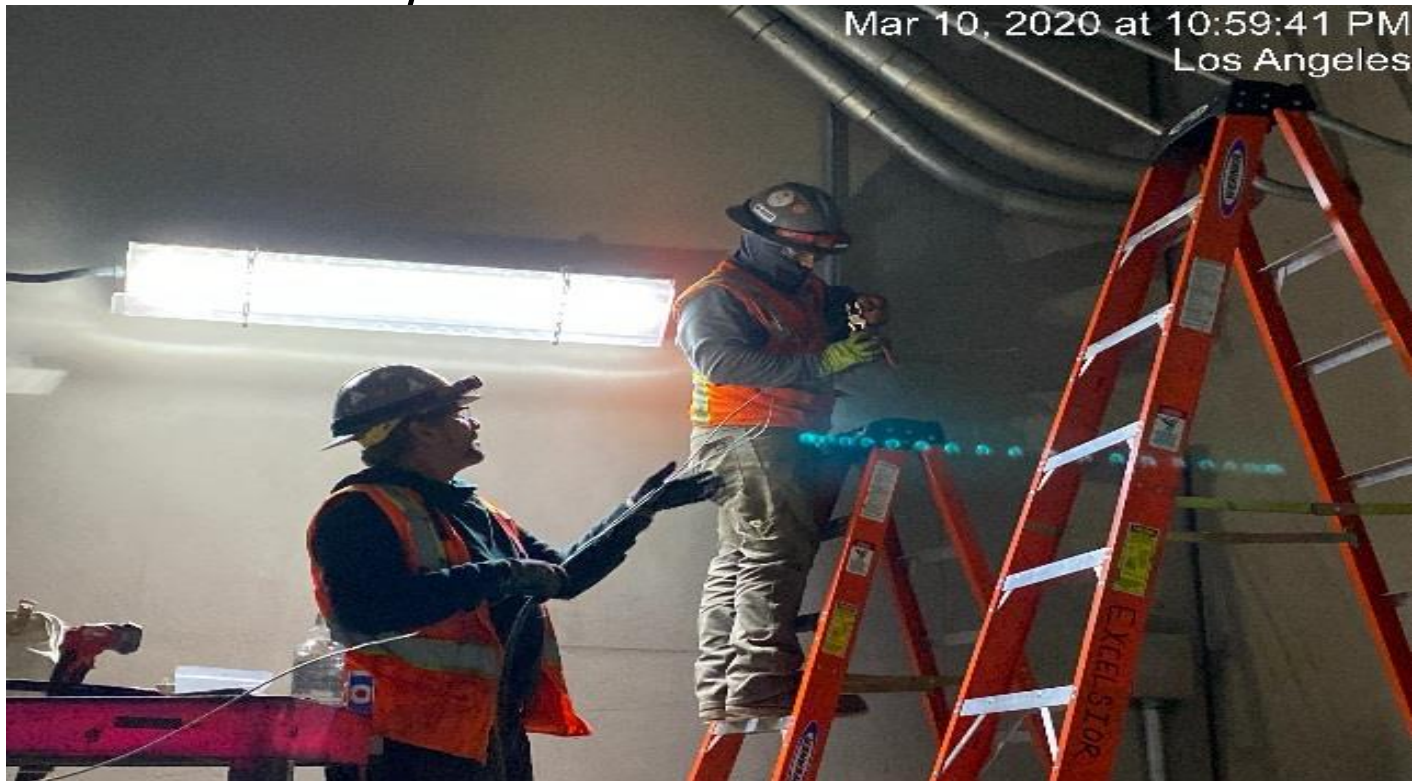
UG-4- – Continue pulling wire for the emergency lighting along the northbound tunnel at Sta 379+00.
