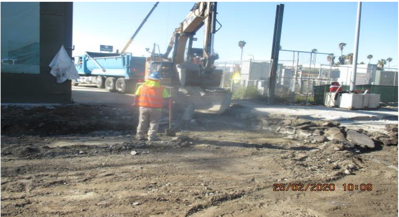
EXPO STATION – Continue demolition/excavation of roadway for new Cul-de-sac entrance on Bronson St. east of the plaza. 2/25/20
