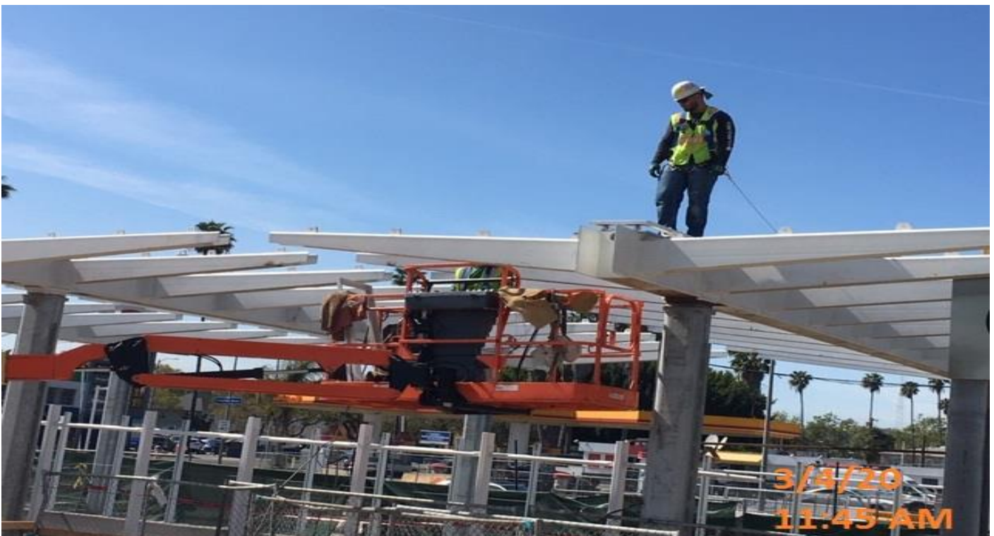
EXPO STATION- Installing cat walk grating above the main entrance canopy structure at the plaza level.
