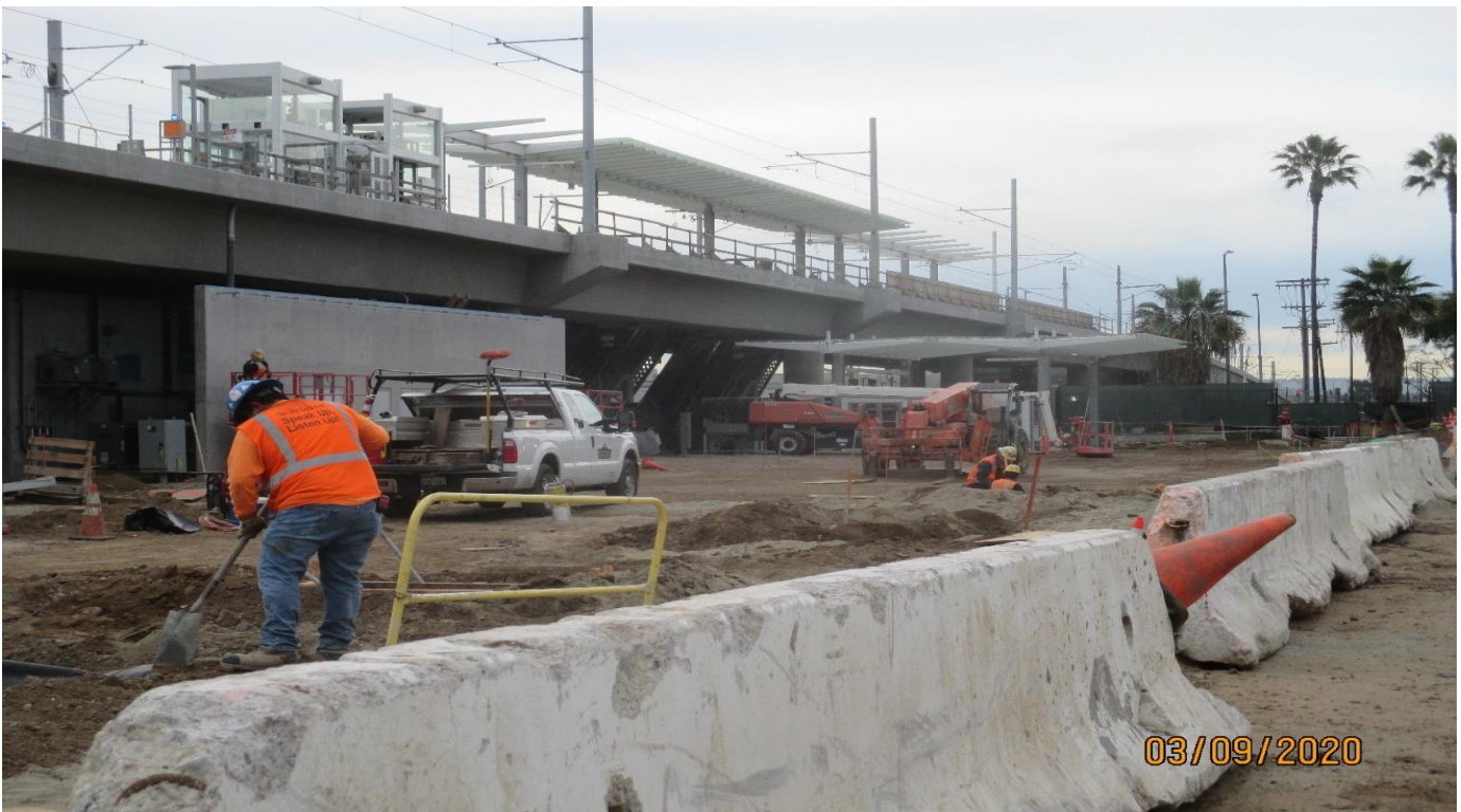
AVIATION/CENTURY- Setting forms and sonatubes for the Aviation Station light pole foundations.
