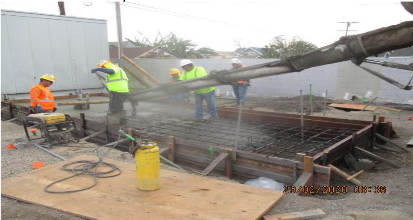
Park Mesa – Placing concrete for the generator pads at TPSS#7 on 60th St & Crenshaw Blvd. 2/29/20
