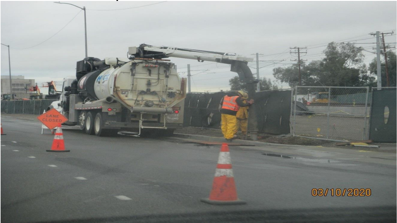
LA BREA – Vacuum truck excavating a light pole foundation at the La Brea Station. Facing west
