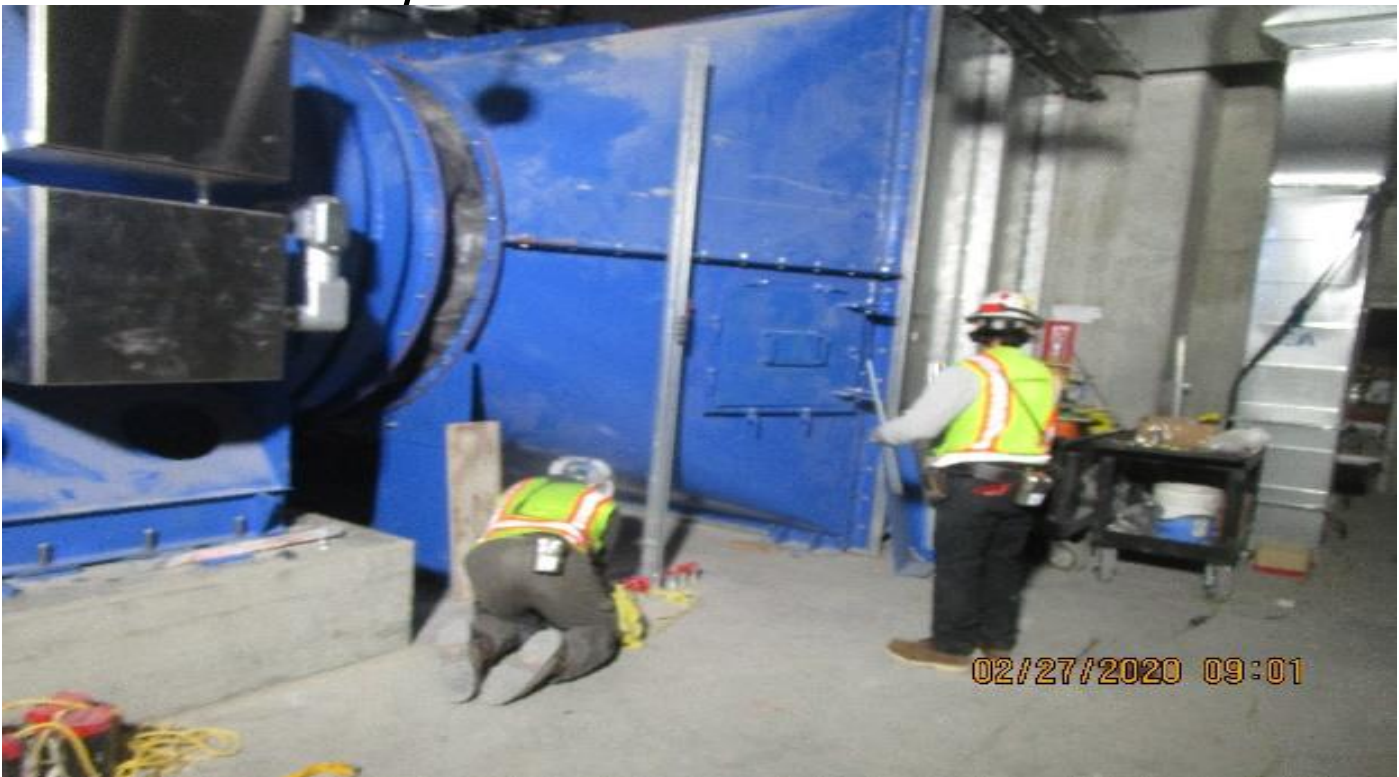
MLK STATION – Rough-in of anchors and supports for the pull box and uni-strut posts for EVF-7-121 in the South Fan Room C – 102 of the concourse level.
