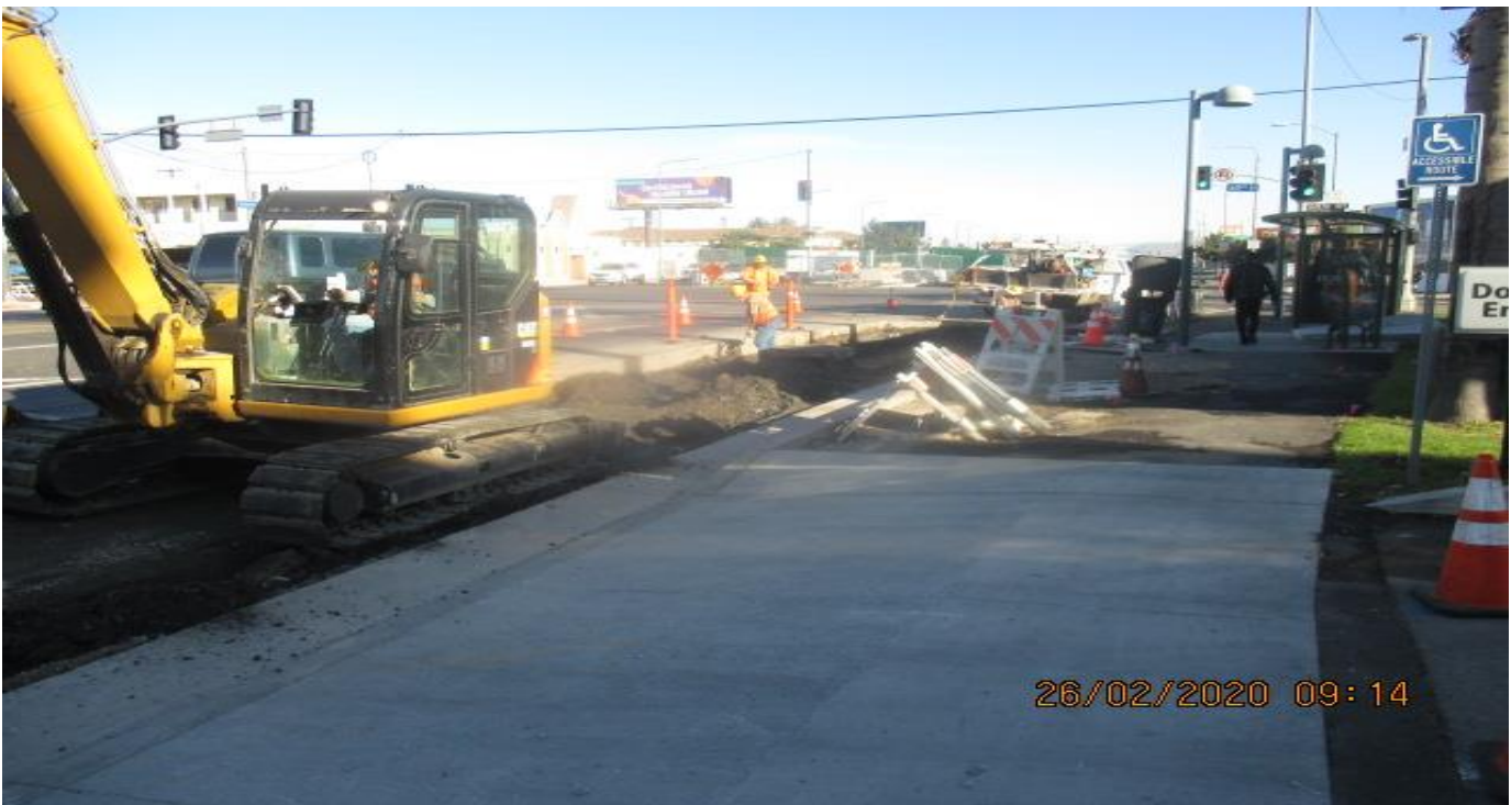
Park Mesa – Continue saw cutting and excavating for bus pad installation on the southeast corner of 60th St & Crenshaw Blvd. 2/26/20
