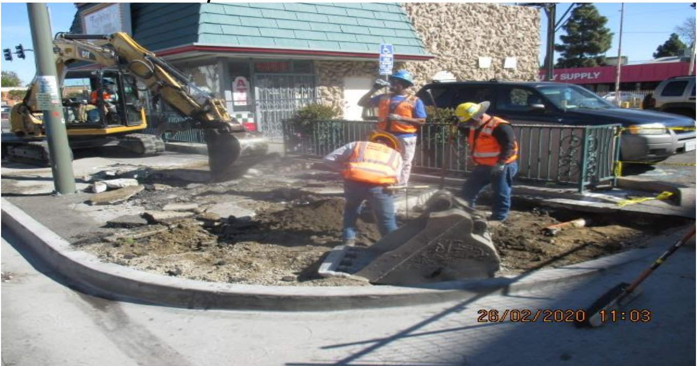
MLK STATION – Saw cutting and excavating for new ADA ramp installation on the southeast corner of Martin Luther King Blvd and Crenshaw Blvd. 2/26/20
