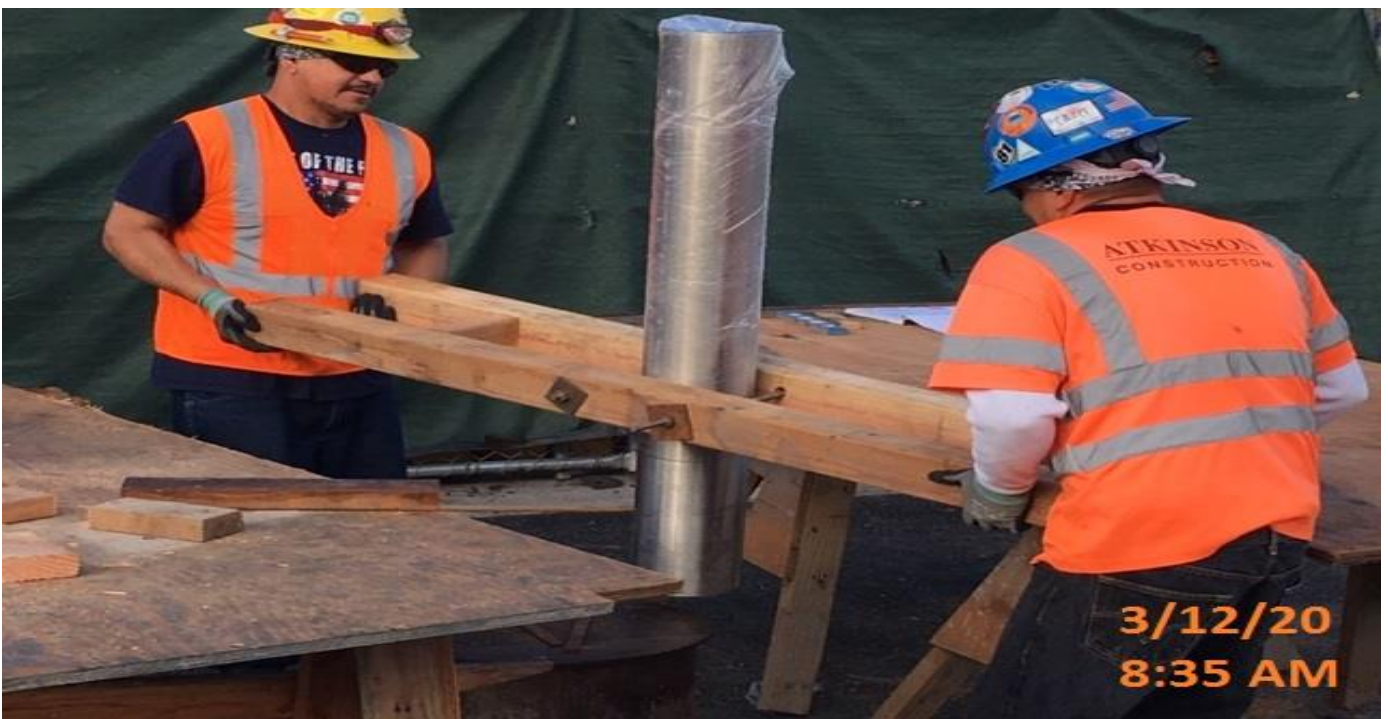
LEIMERT PARK STATION – Fabricating stainless steel station bollards at the plaza level.
