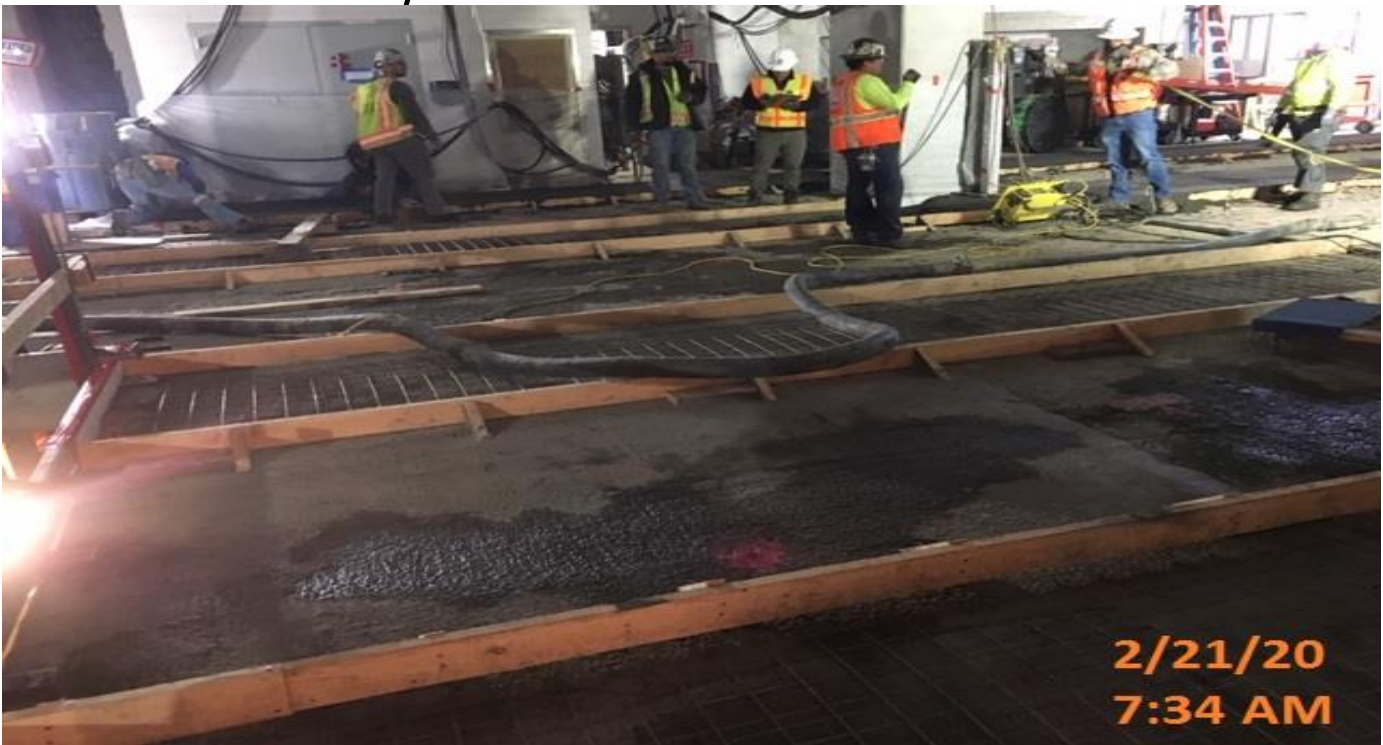
MLK STATION – Placing 1st phase of concrete on the architectural topping slab at the concourse level.
