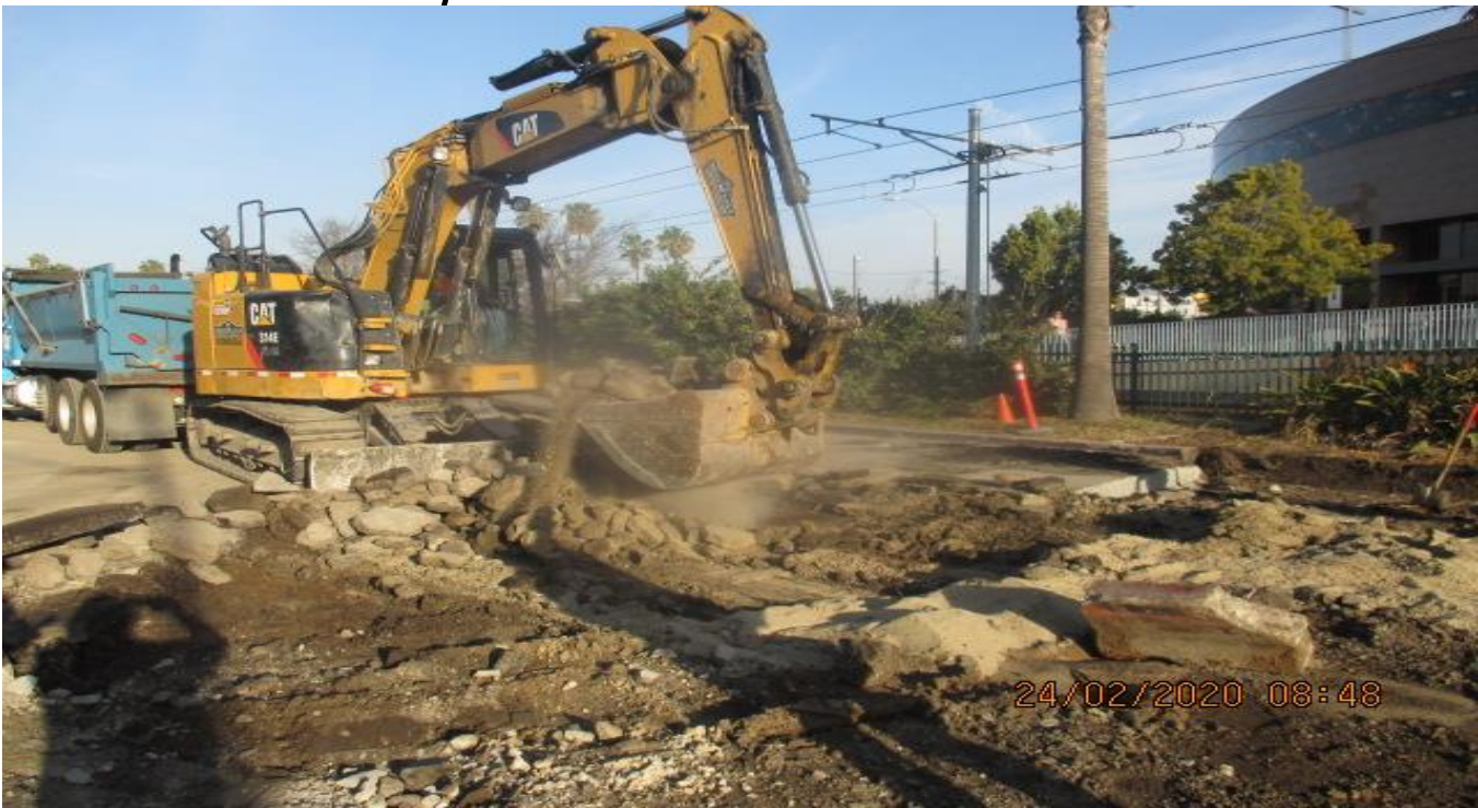
EXPO STATION – Continue demolition/excavation of roadway for new Cul-de-sac entrance on Bronson St. east of the plaza. 2/24/20
