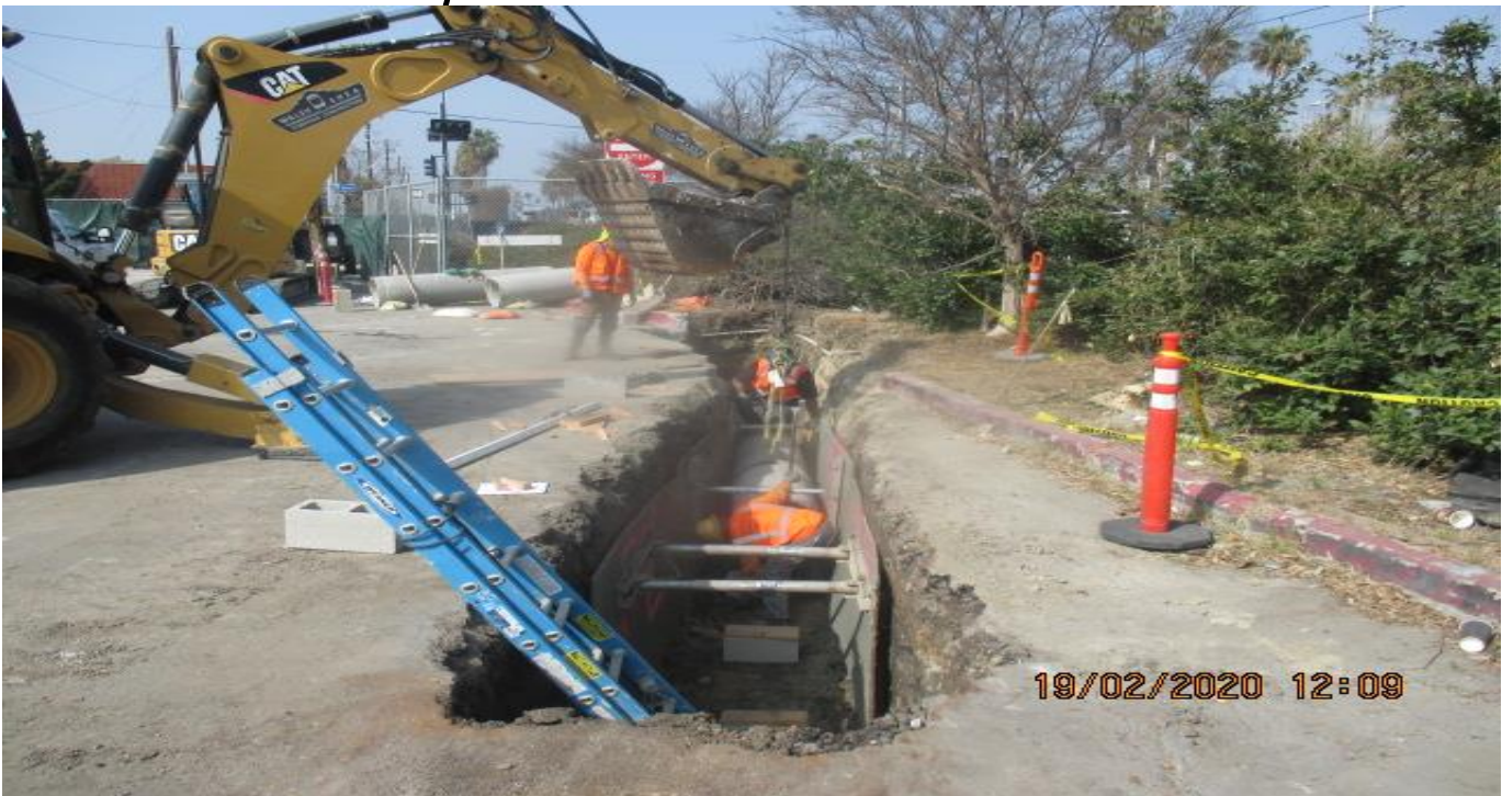
EXPO STATION – Installing sections of 18” RCP for Line B – storm drain at the Cul-de-sac on Bronson St. east of the plaza. 2/19/20
