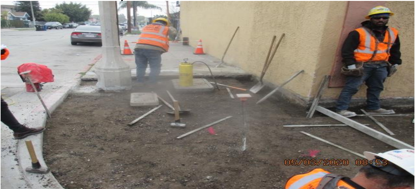
Park Mesa – Installing block-out forms in preparation for new concrete placement of sidewalk and ADA ramp on the southeast corner 63rd St and Crenshaw Blvd. 3/5/20
