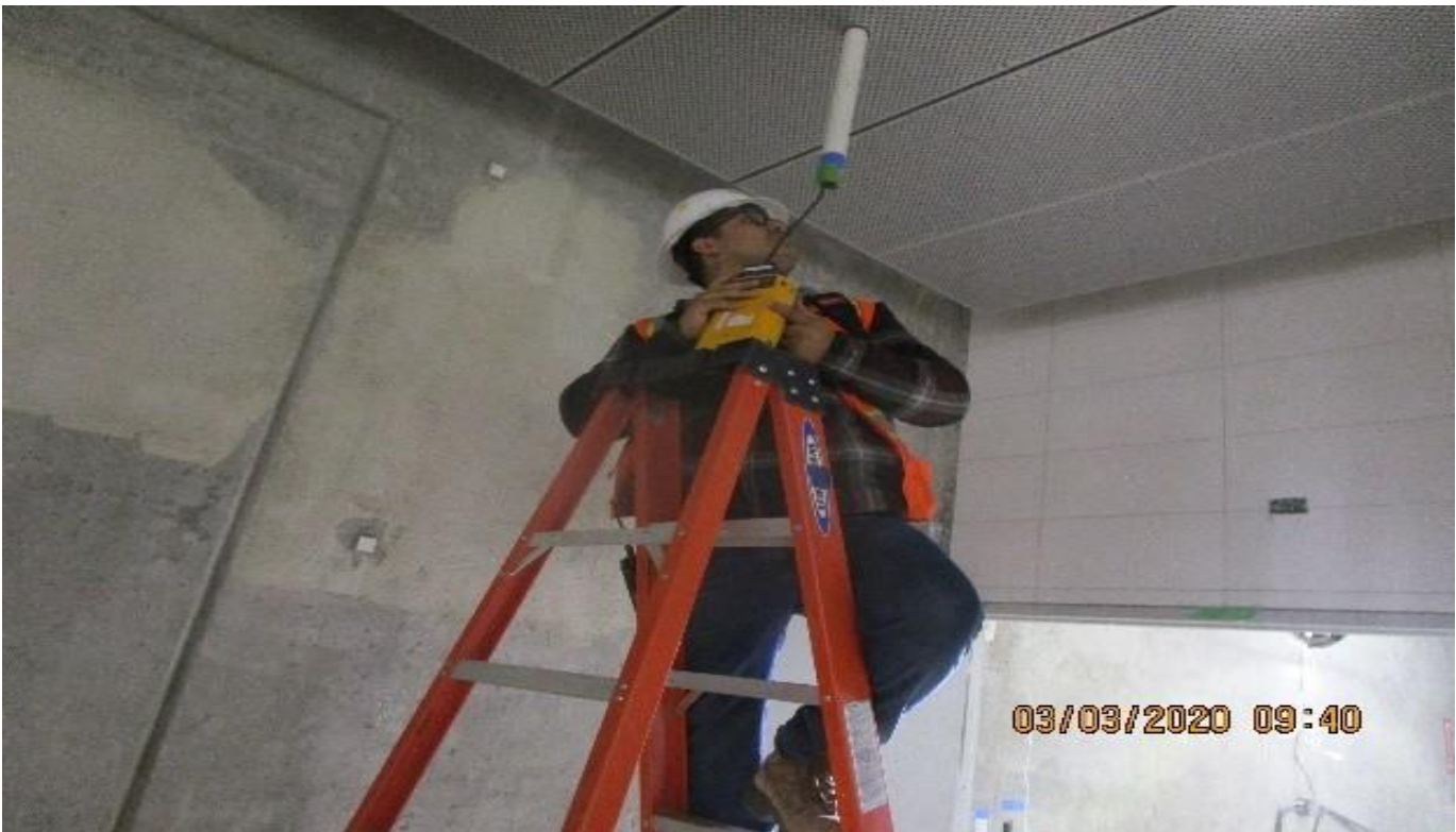
MLK STATION – Free Area C118 & Paid Area C119, Begin at device locations continuity testing CAT-6 cables for LCD-CCTV.
