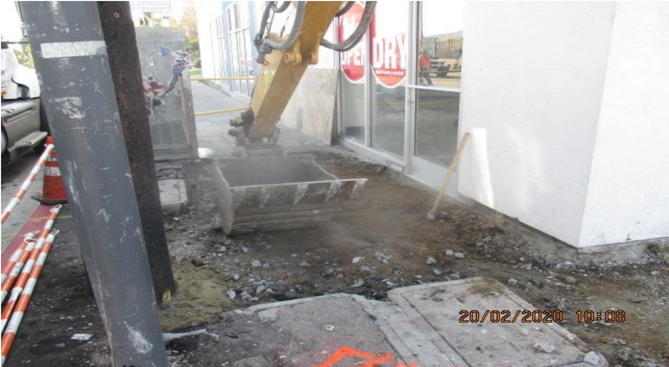
Park Mesa – Excavating/backfill for new sidewalk and ADA ramp installation on the southeast corner of Hyde Park Blvd and Crenshaw Blvd. 2/20/20
