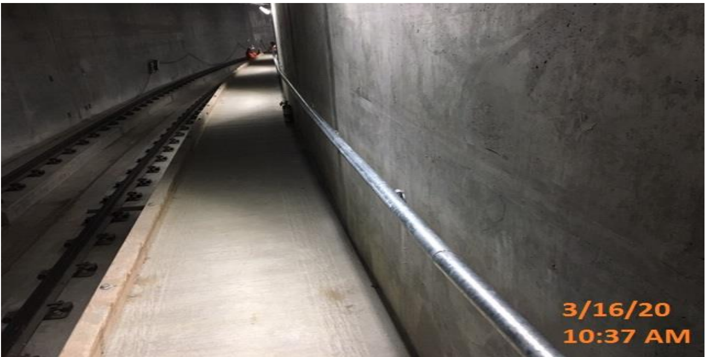
UG3 – Installing handrails for the emergency walkway throughout the north and southbound tunnels.
