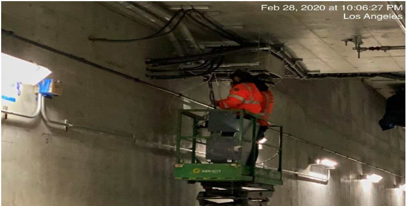
UG3 – Continued slicing wire to tunnel booster junction boxes in the northbound tunnel at Sta 291+50.
