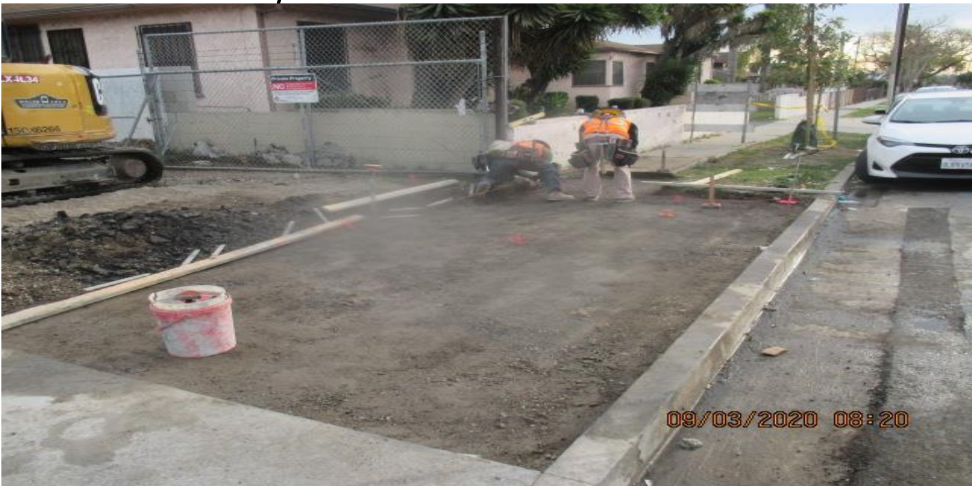
Park Mesa – Building block-out forms for the new sidewalk/driveway installation for TPSS#7 entrance on 60th St & Crenshaw Blvd. 3/9/20
