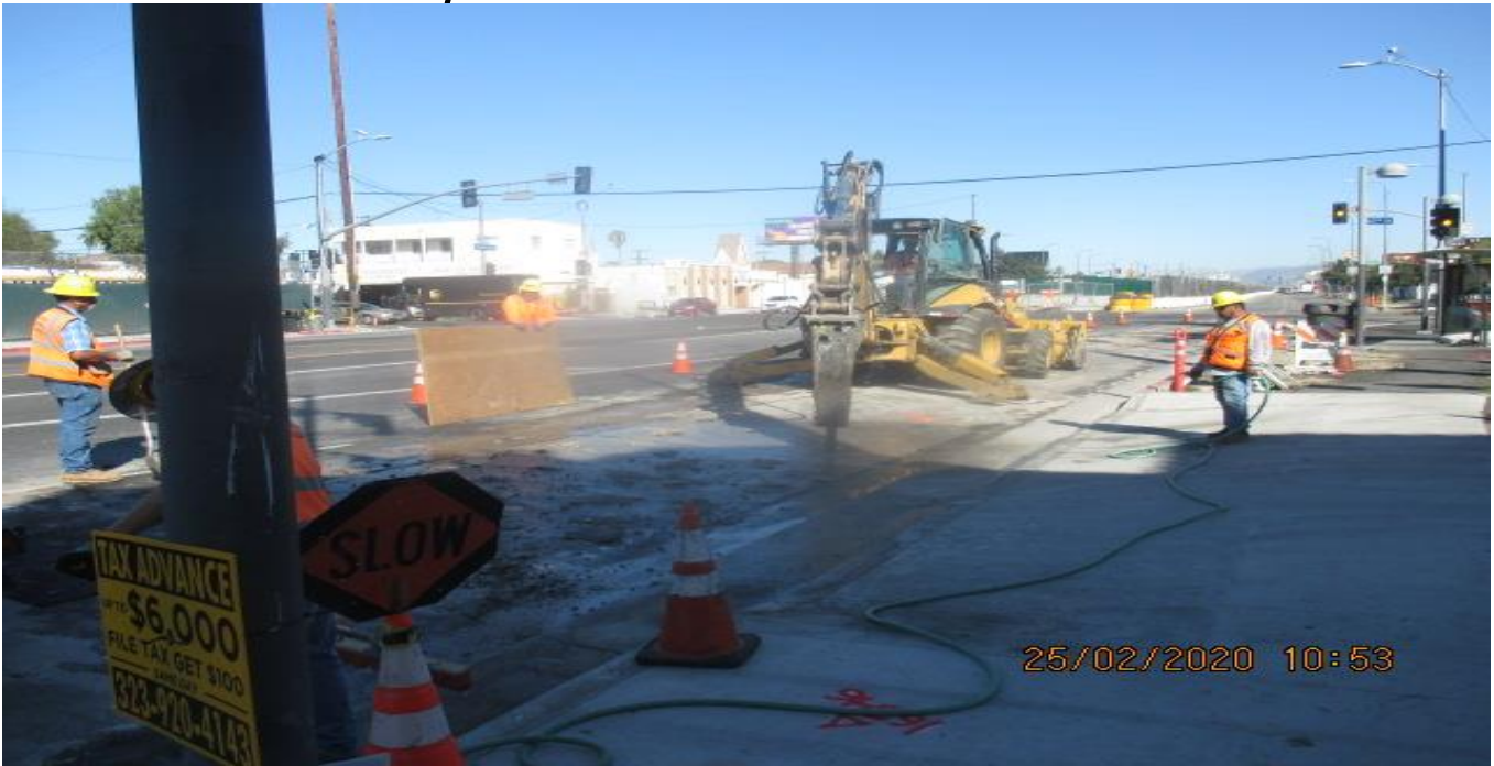
Park Mesa – Saw cutting and excavating for bus pad installation on the southeast corner of 60th St & Crenshaw Blvd. 2/25/20
