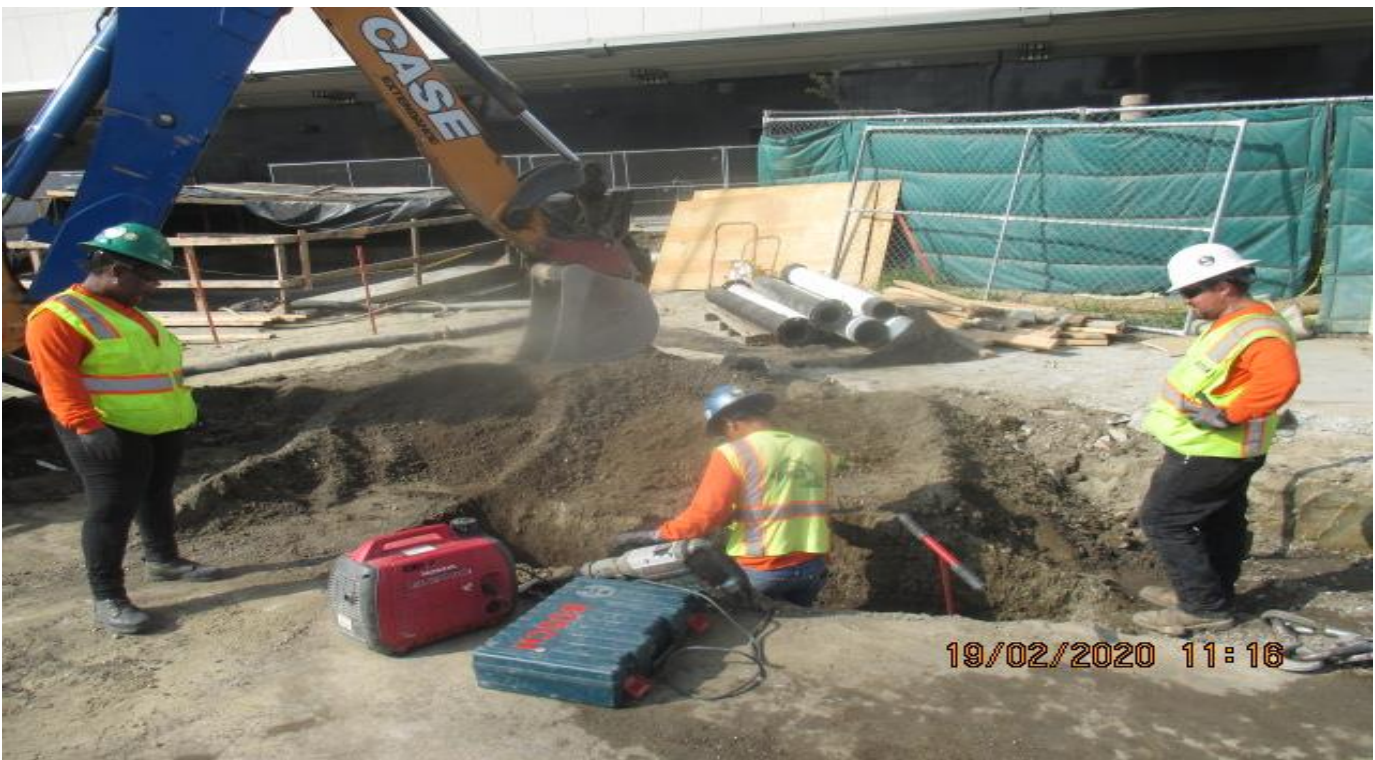
MLK STATION – Excavating for LADWP fire water service connection for entire station at the plaza level. 2/19/20
