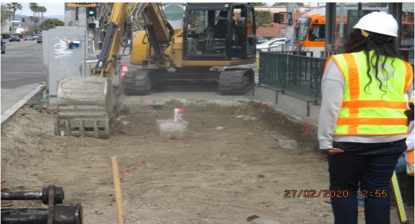
MLK STATION – backfilling/compacting for new sidewalk and ADA ramp installation on the southeast corner of Martin Luther King Blvd and Crenshaw Blvd. 2/27/20
