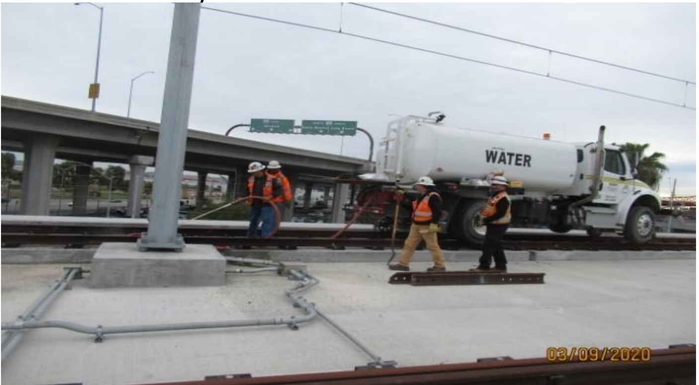
GUIDEWAY - HCC on NB1300 track east leg of Wye removing debris from bridge deck (looking east)
