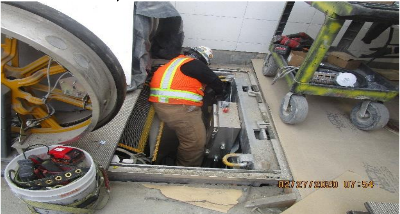
LEIMERT PARK STATION – Installing conduit to junction boxes for Escalators 1&2 at the intermediate level.
