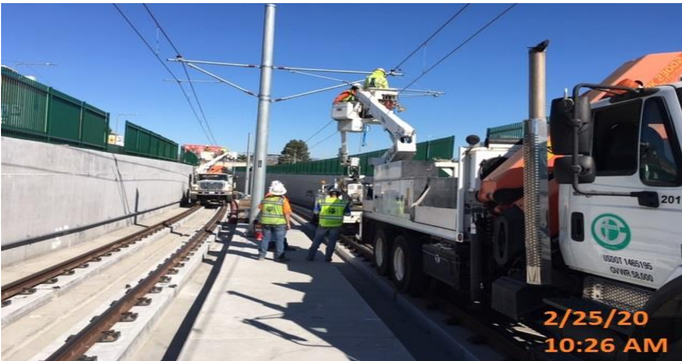
UG4 – Registering and staggering guide sections for the overhead contact system poles at the south end portal.
