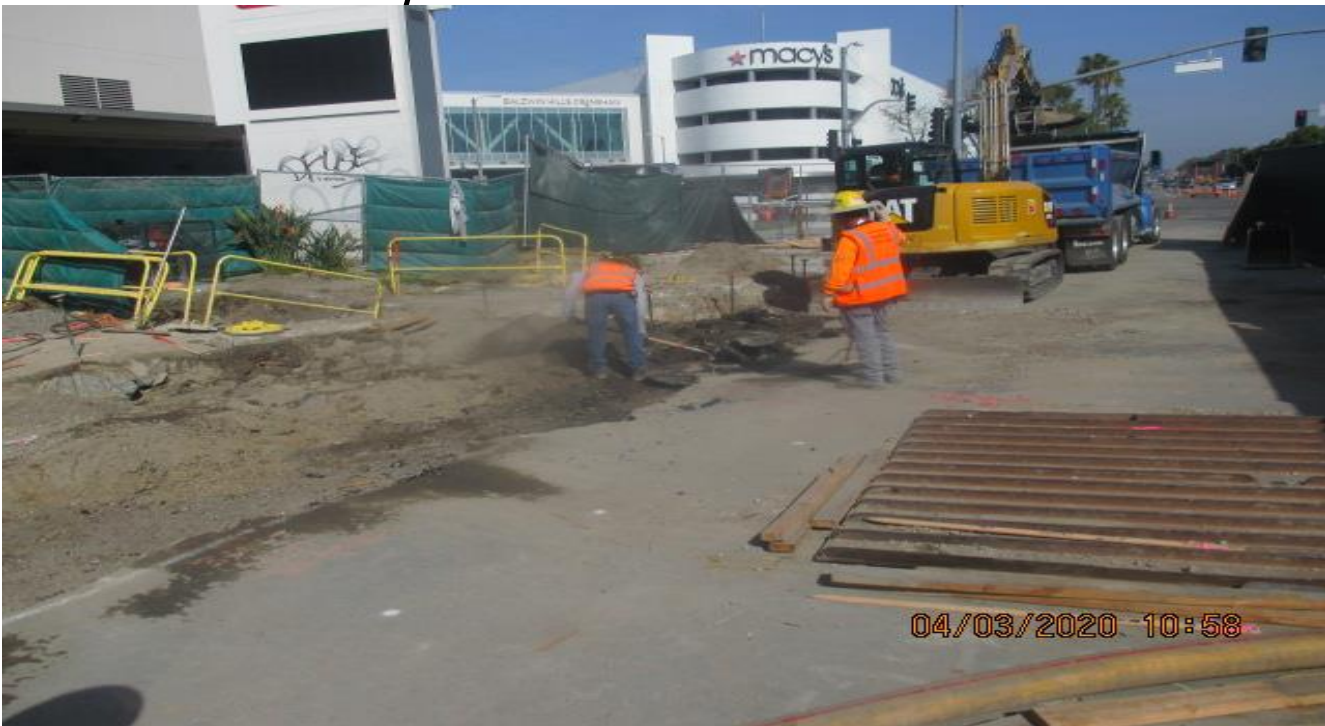
LEIMERT PARK STATION – Excavating for new curb/gutter and sidewalk installation on the southwest corner of Martin Luther King Blvd and Crenshaw Blvd. 3/4/20
