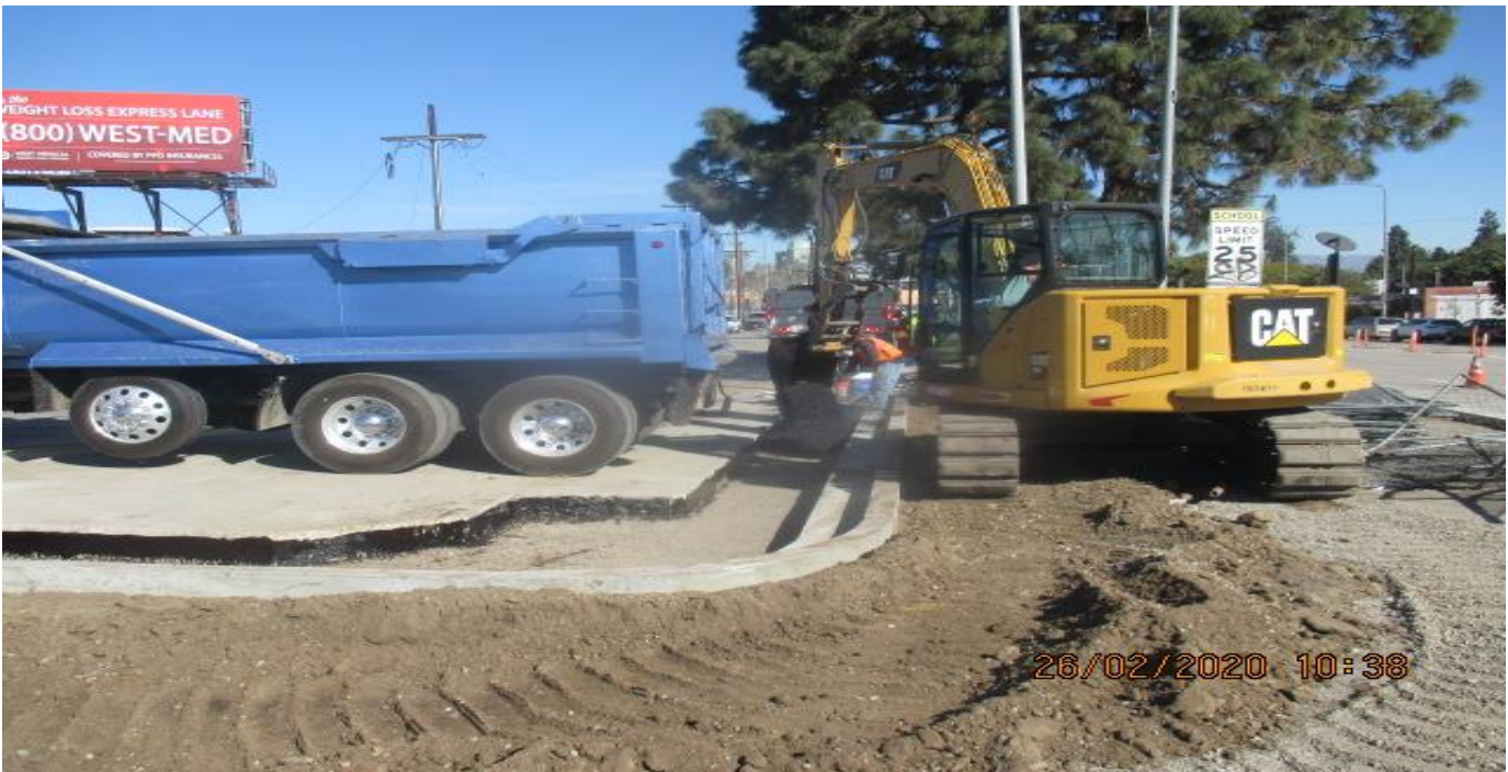
LEIMERT PARK STATION – Placing asphalt concrete and compacting sidewalk on northbound Leimert Blvd and Crenshaw Blvd. 2/26/20
