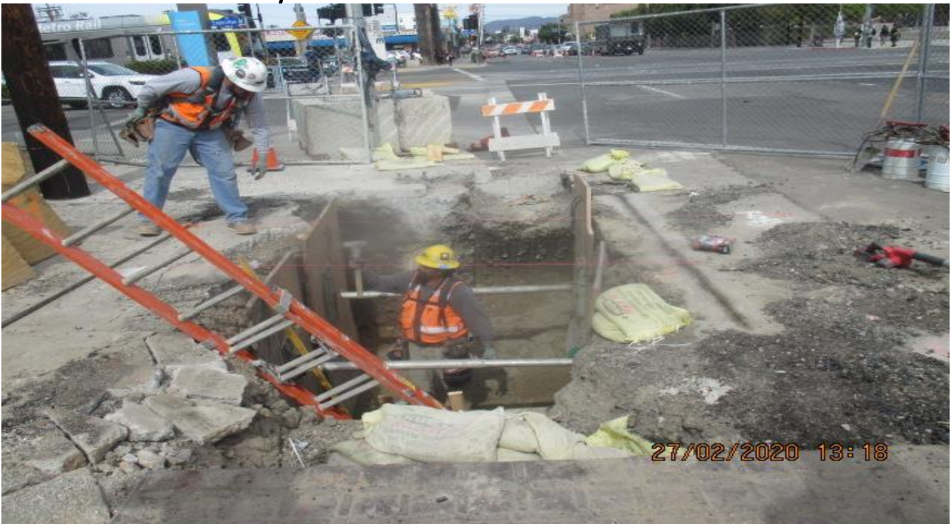
EXPO STATION- Building steam wall forms for Catch Basin #19 on the northeast corner of Exposition Blvd and Crenshaw Blvd. 2/27/20
