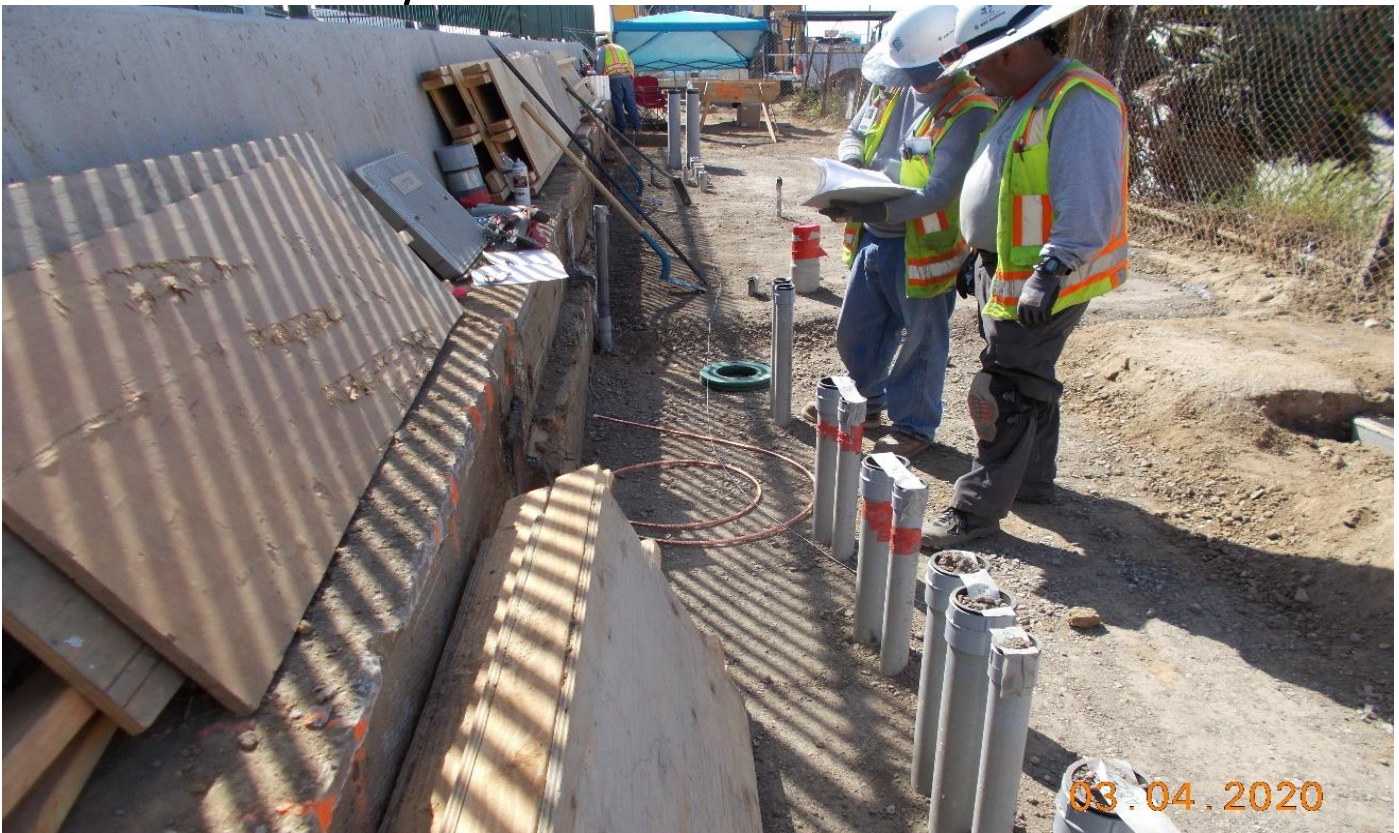
104th STREET – 104th St - Dyna Electric pulling string lines in MCC conduits.
