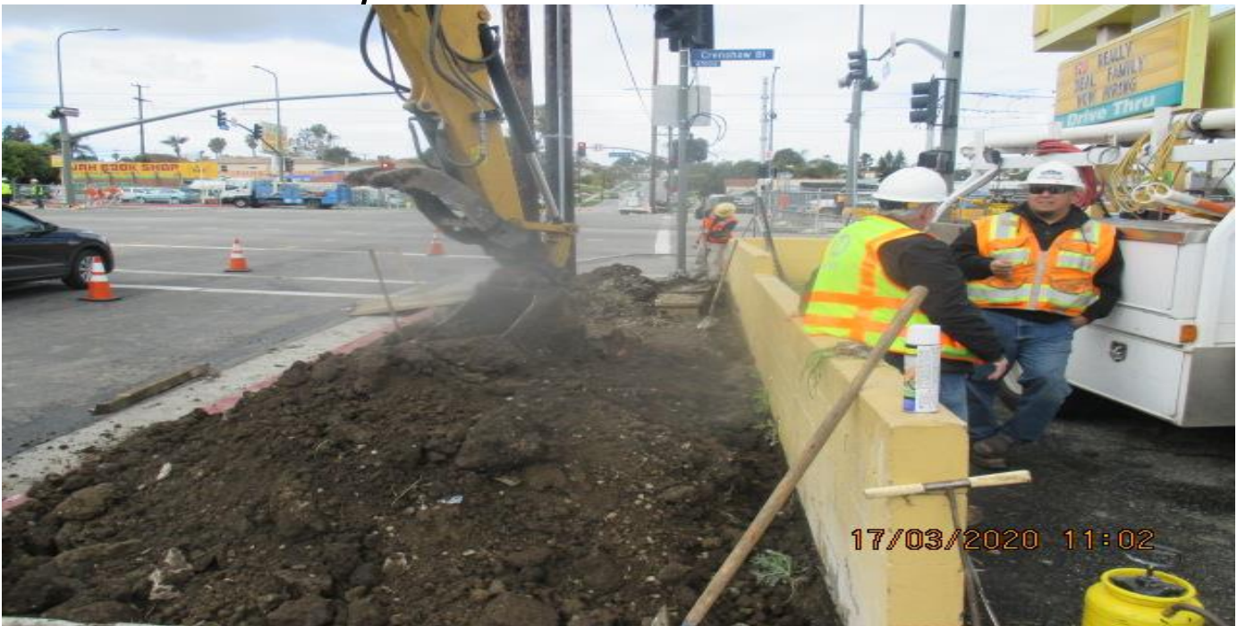
Park Mesa – Excavating/demolishing for new concrete sidewalk installation on the northeast corner of 48th St and Crenshaw Blvd. 3/17/20
