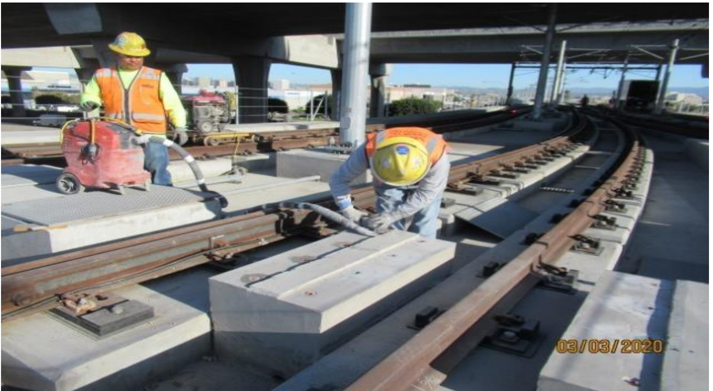
GUIDEWAY - WSCC hand grinding epoxy on concrete foundation for west leg of Wye STA 13+01
