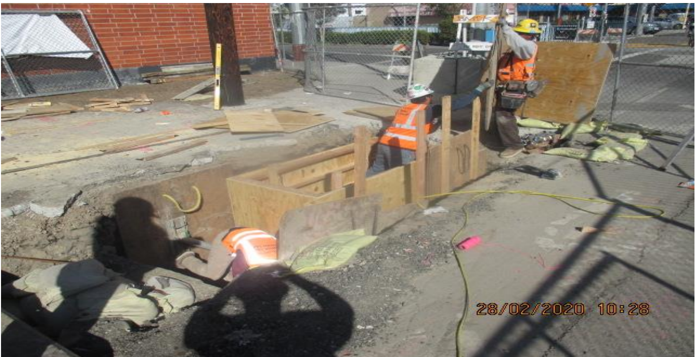
EXPO STATION- Continue building steam wall forms for Catch Basin #19 on the northeast corner of Exposition Blvd and Crenshaw Blvd. 2/28/20
