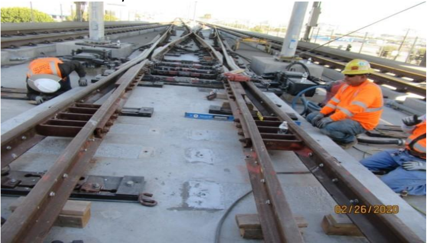
GUIDEWAY - WSCC checking plane on surface for concrete MPF at GL Wye STA 13+90 (looking north) Rework
