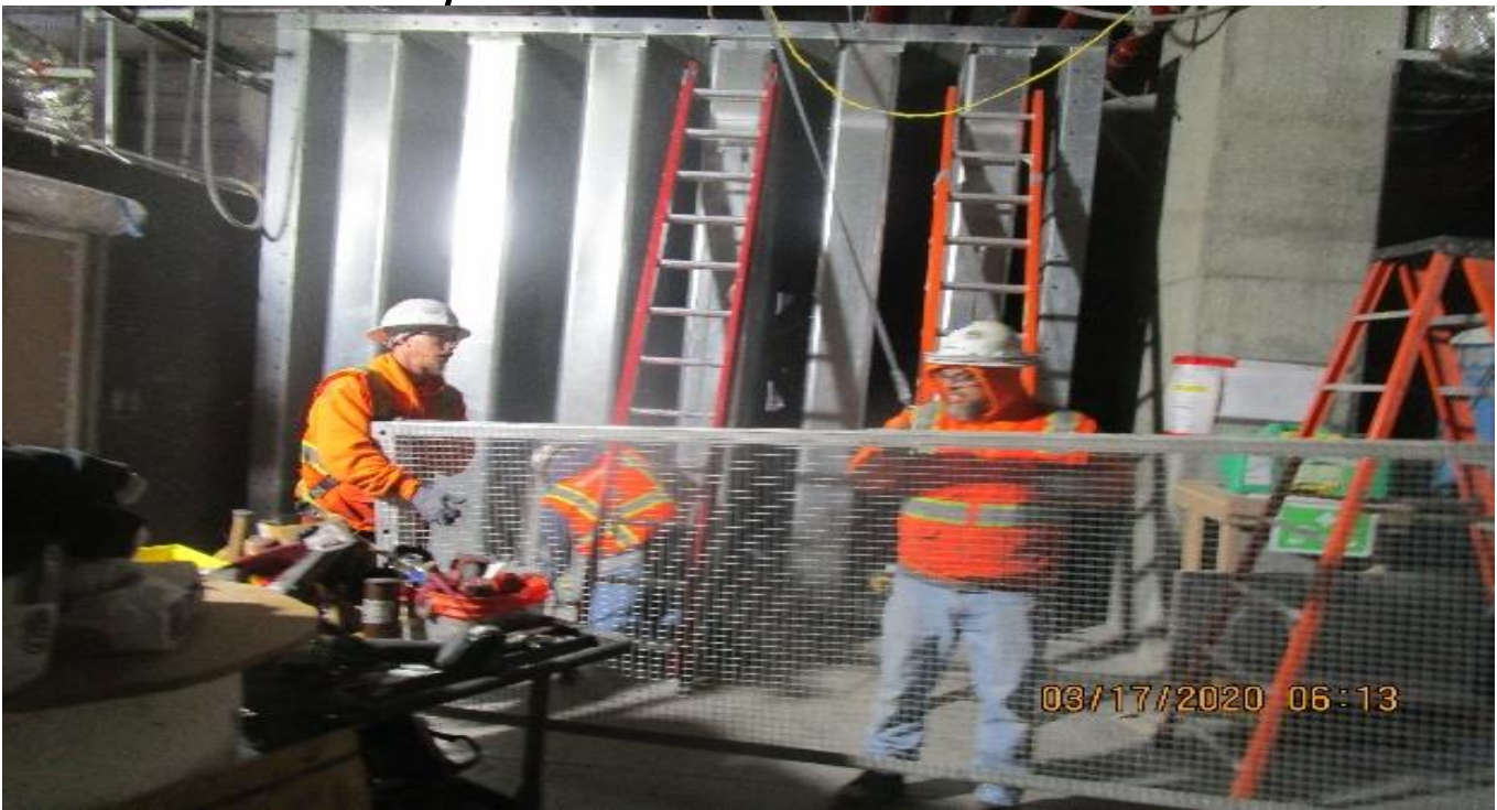
LEIMERT PARK STATION – Installing bird protection screens on the sound attenuators for EVF-6-302 in the North Fan Room C – 142 of the concourse level.
