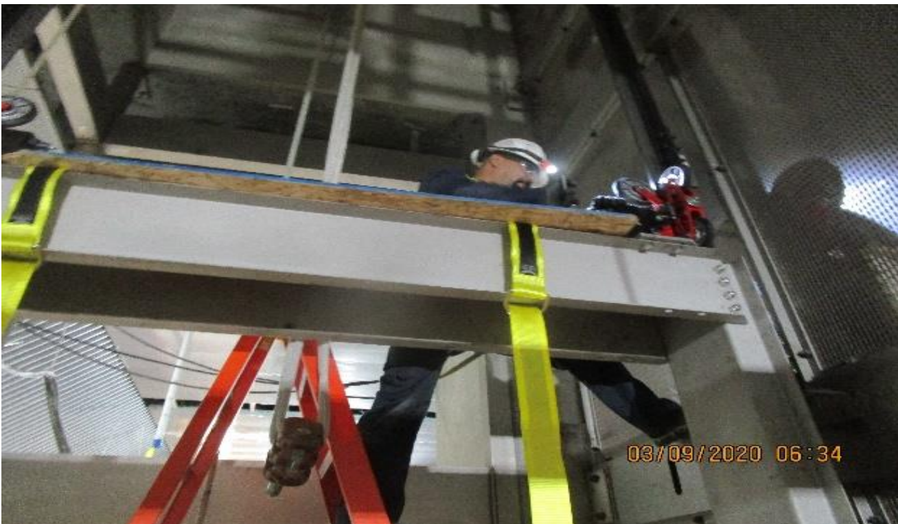
LEIMERT PARK STATION – Continue aligning hoist way guide rails and rollers for Elevator Structures 3&4 at the platform level.
