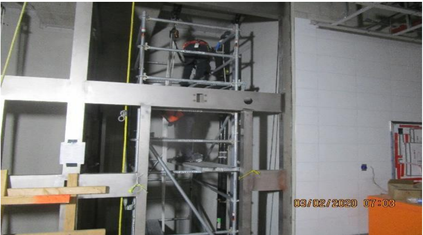
LEIMERT PARK STATION – Continue guide rail bracket support for Elevator hoist way/pit 3 at the concourse level. 3/2/20
