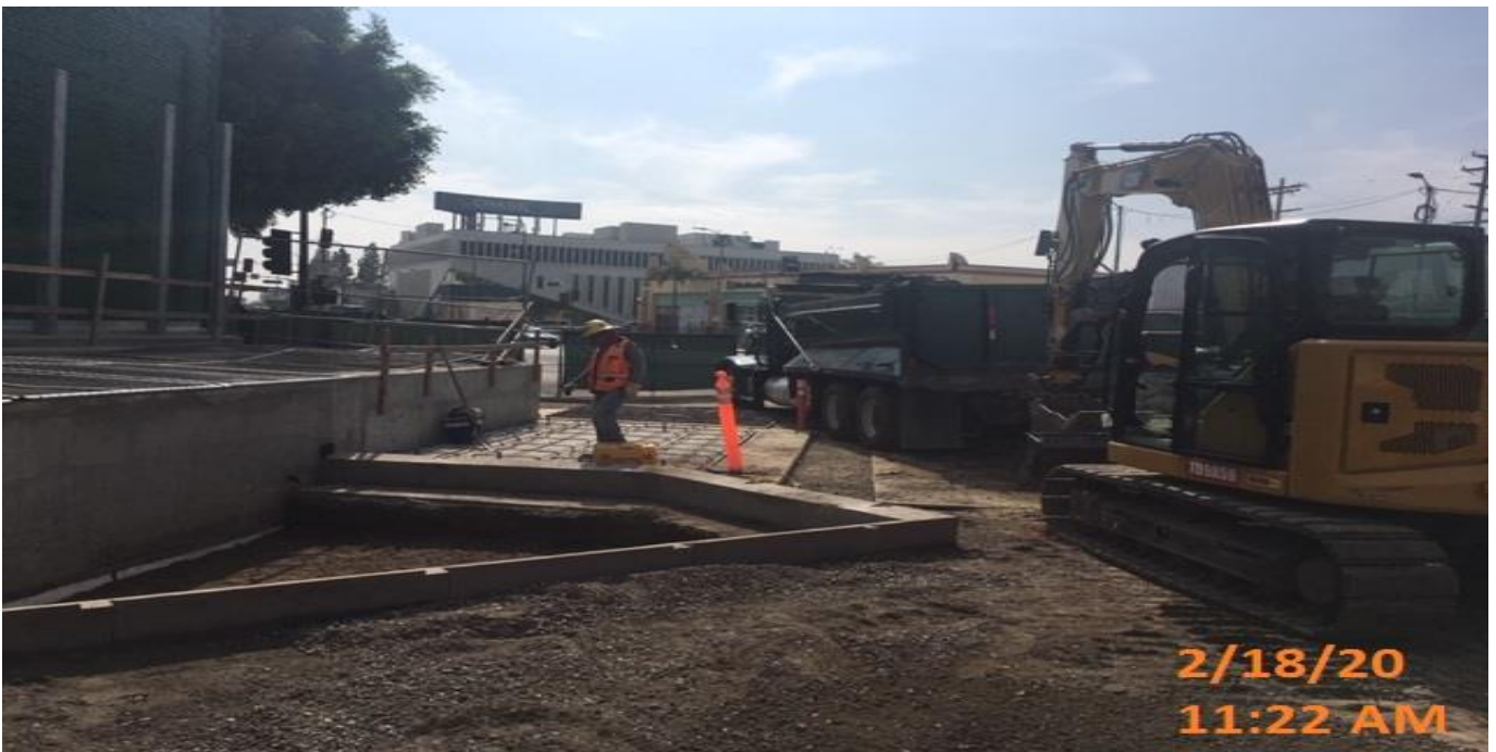
LEIMERT PARK STATION – Continue excavating for planar wall sections at the northeast end of the plaza level.
