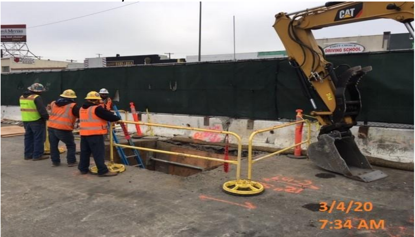
MLK STATION – WSCC crew and Norcal continue exploratory work on leak repair.
