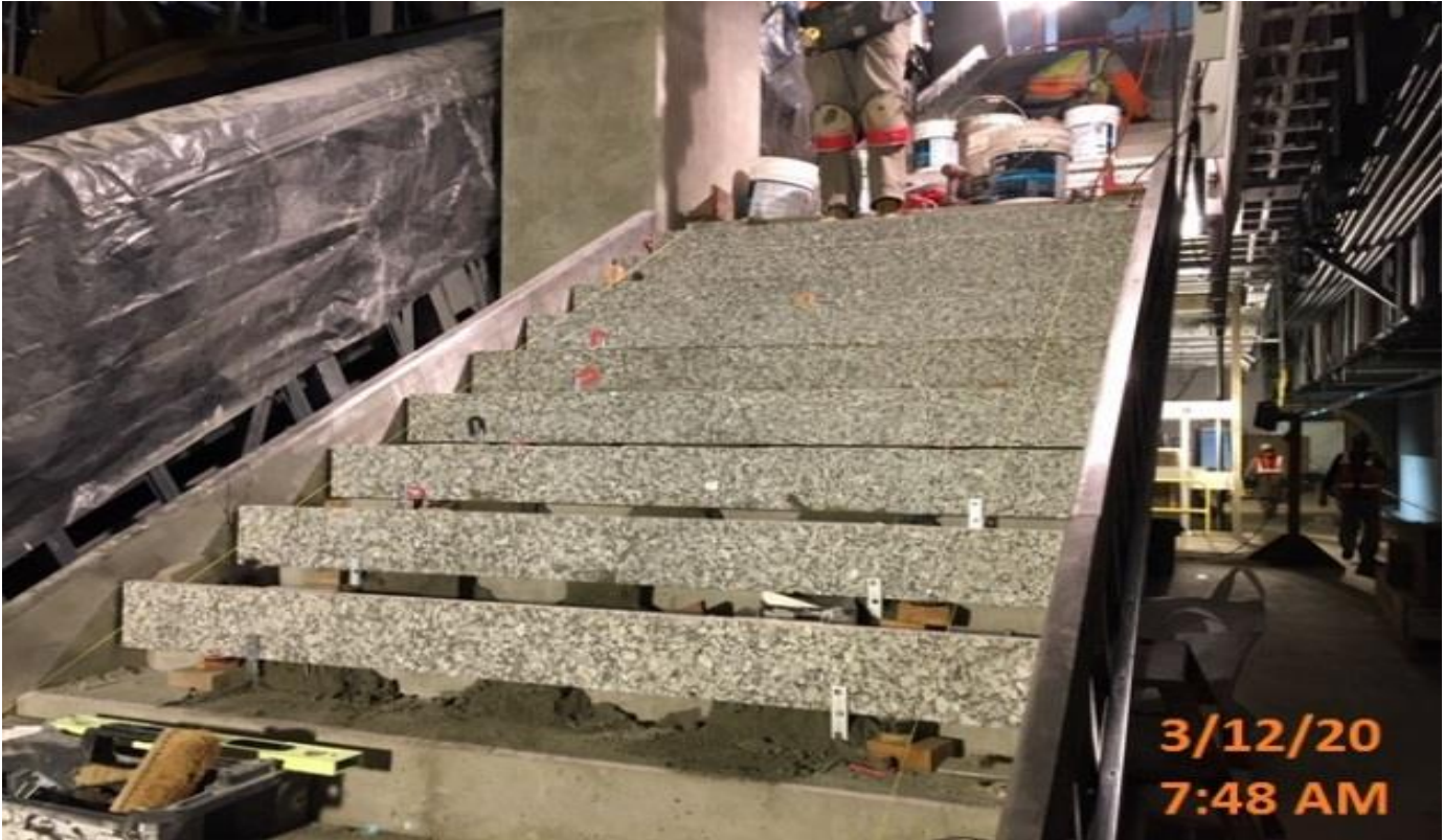
MLK STATION - Began granite riser installation for staircase#3 at the concourse level.
