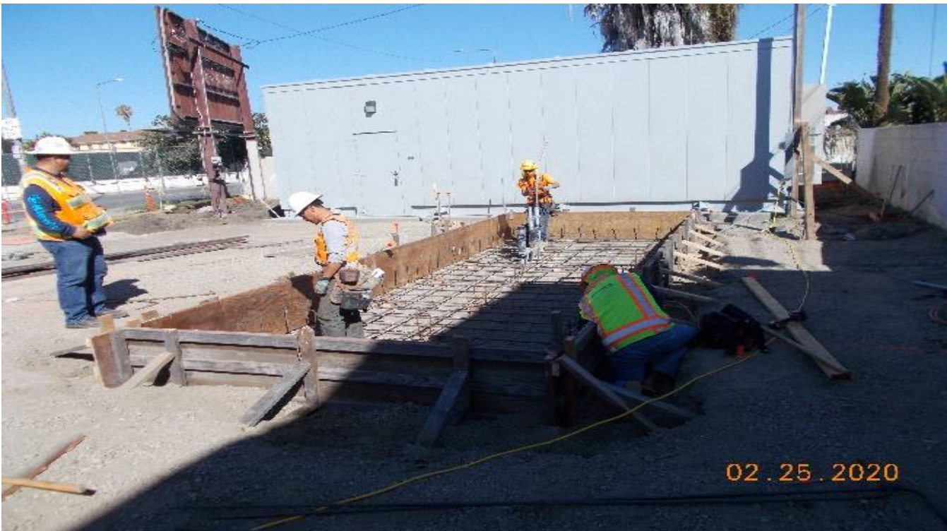
Park Mesa – Began formwork and rebar installation for the generators at TPSS#7 on 60th St & Crenshaw Blvd.
