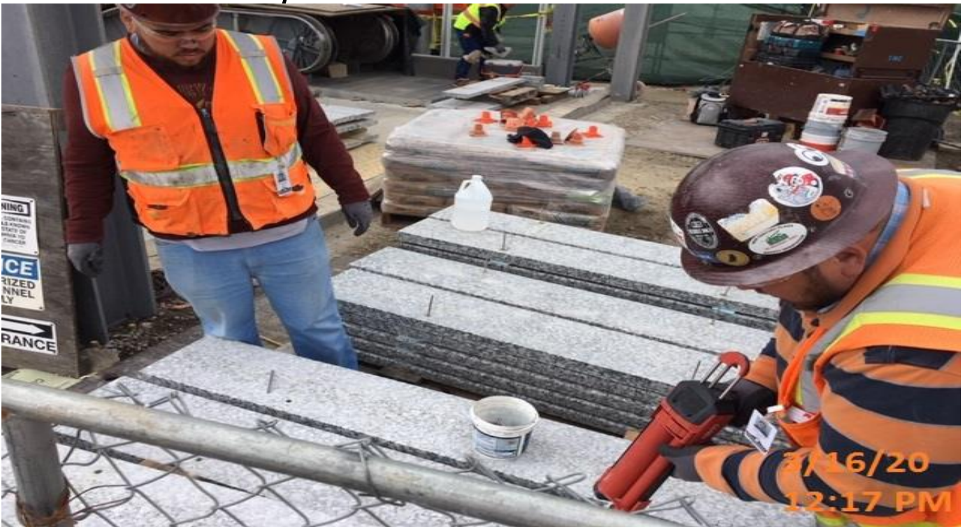
EXPO STATION- Continue installing granite risers at the main entrance staircase landing of the plaza level.
