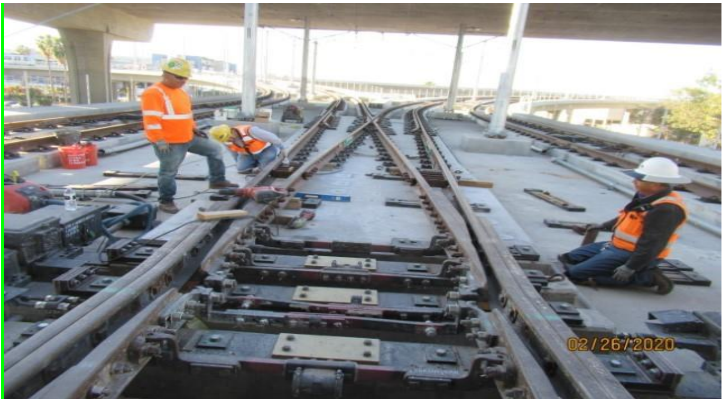
GUIDEWAY - WSCC preforming repair work on concrete slab for even surface under fasteners MPF STA 13+90 GL Wye.
