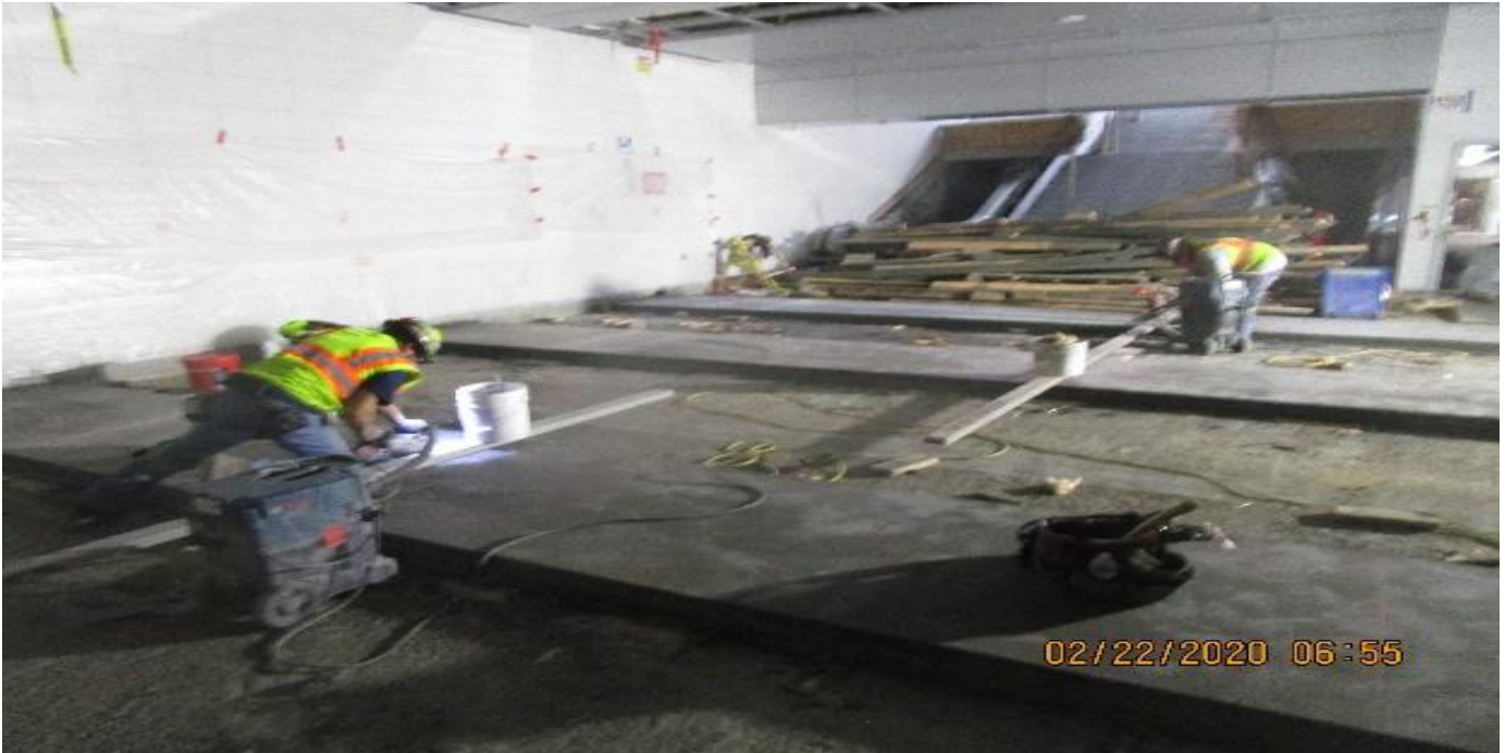
MLK STATION – Saw cut for expansion joints and buffing the architectural topping slab at the concourse level.
