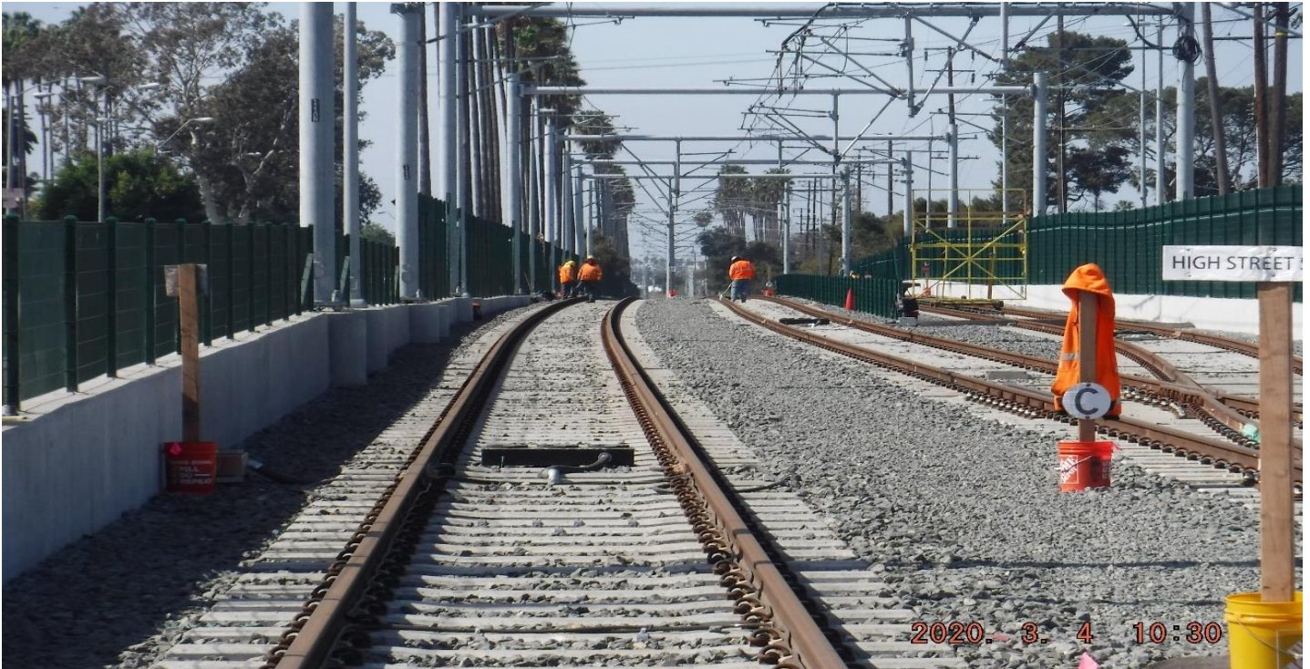
Florence/Ivy - STA256+10_ Looking North_ Disturbed track structure OCS#1212_ PUNCH LIST_ High.
