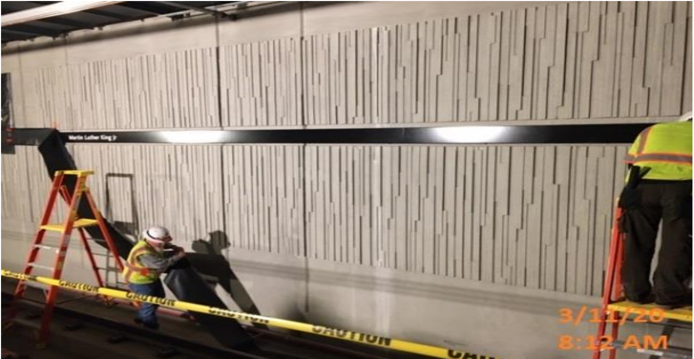
MLK STATION - Completing installation of the Metro signage at the platform level.
