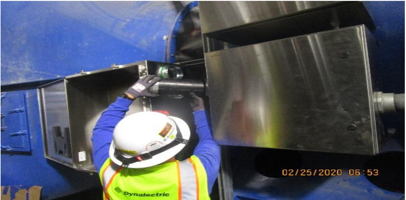
LEIMERT PARK STATION – Continue installing conduit to the pull box for EVF-6-101 in the South Fan Room C – 102 of the concourse level.
