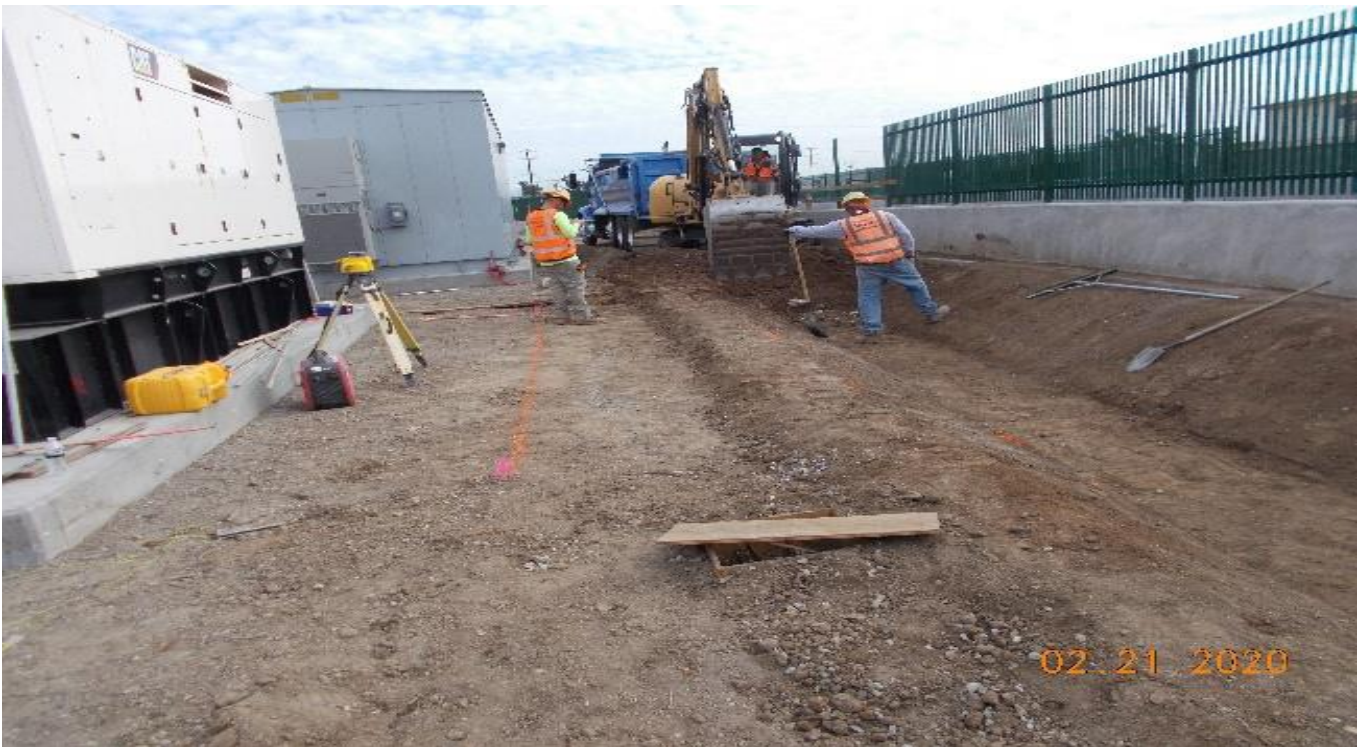
UG3 – Continue excavation for culvert drainage along the southbound barrier wall from Sta 279
