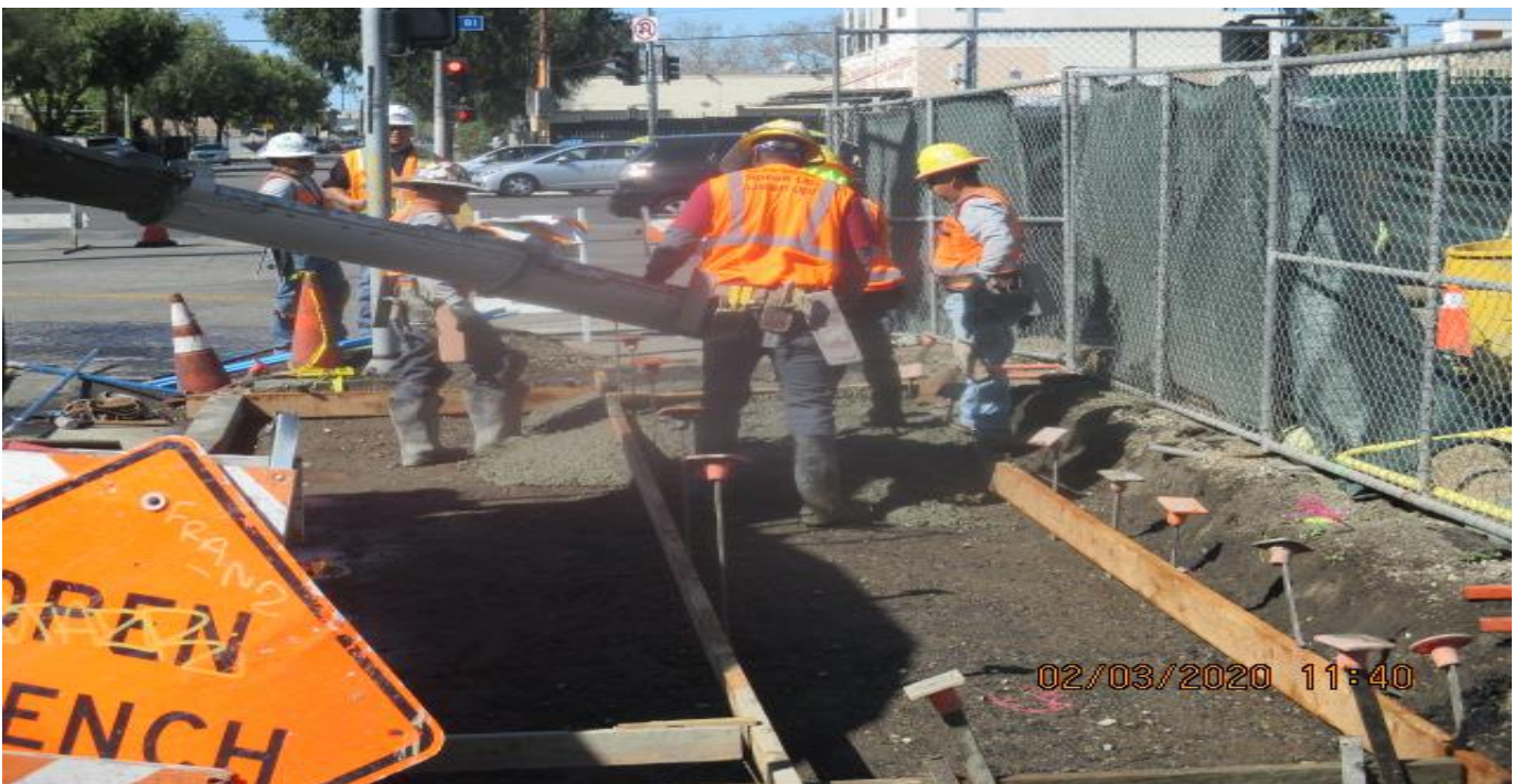
Park Mesa – Installing block-out forms and placing concrete for sidewalk/driveway for TPSS#7 entrance on 60th St & Crenshaw Blvd. 3/2/20
