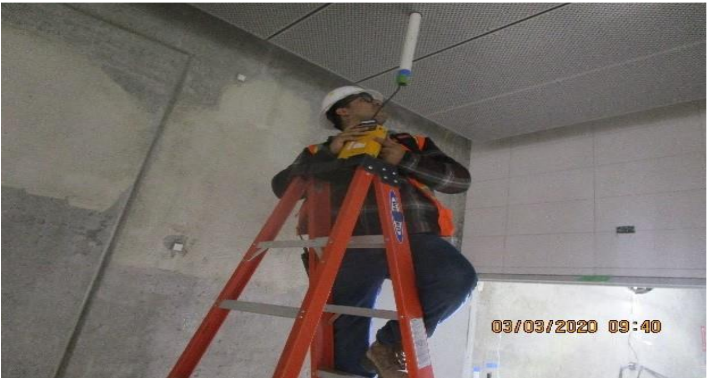
MLK STATION – Free Area C118 & Paid Area C119, Begin at device locations continuity testing CAT-6 cables for LCD-CCTV.
