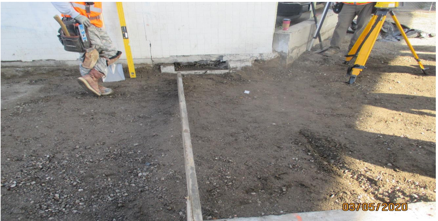
MANCHESTER AVE- Drain that was forgotten and need to be placed in the sidewalk on Manchester.
