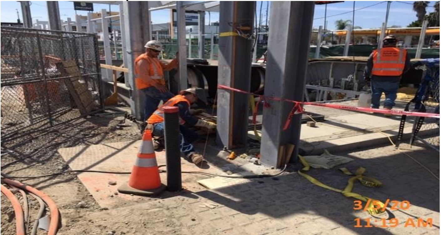
EXPO STATION- Welding frame for the emergency exit stairs at the main entrance of the plaza level.
