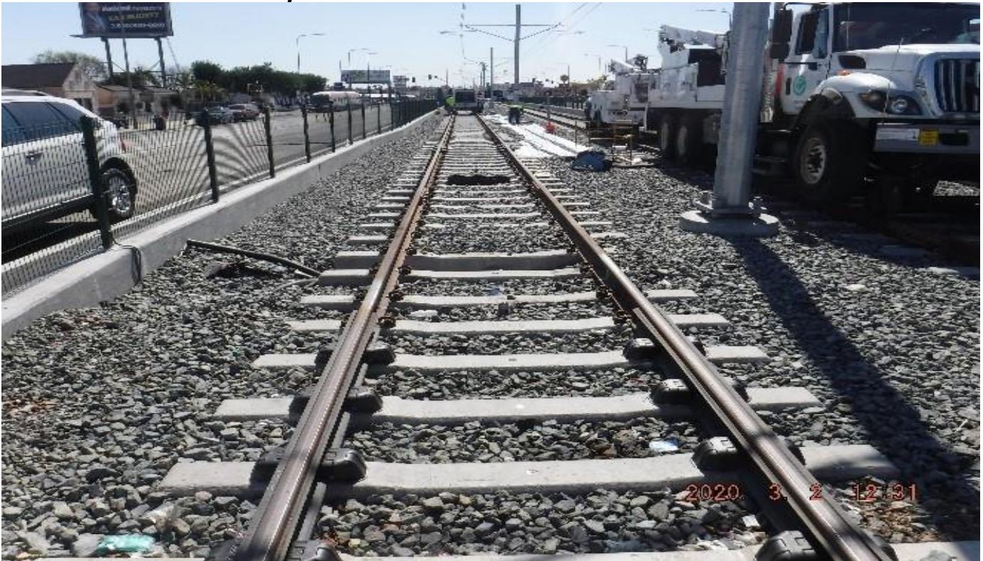
SLAUSON STA – STA 330+00 TK#4-NB looking south – placing cables in duct bank between Slauson Ave and 57th St.
