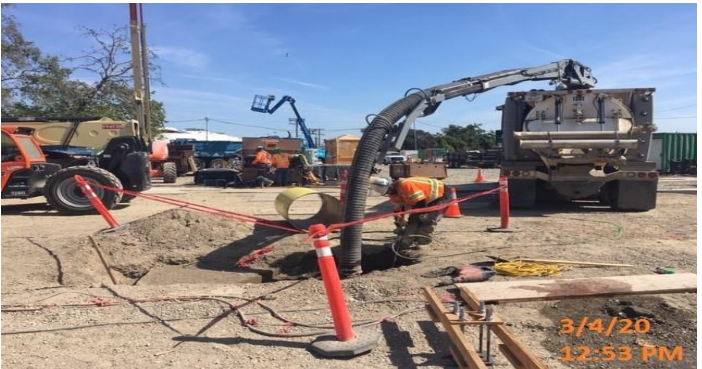
EXPO STATION- WSCC crew potholing and setting sono tubes for plaza lighting
