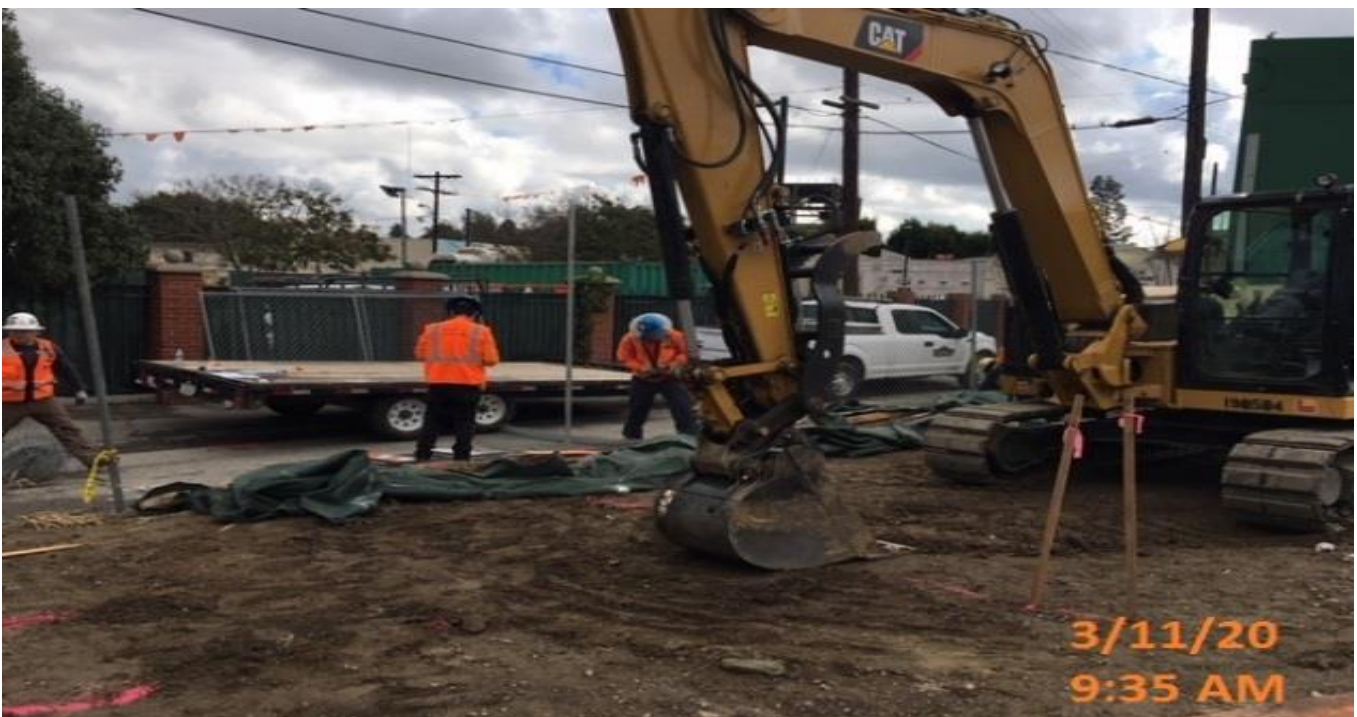
LEIMERT PARK STATION – Began excavating for the east emergency exit staircases at the plaza level.
