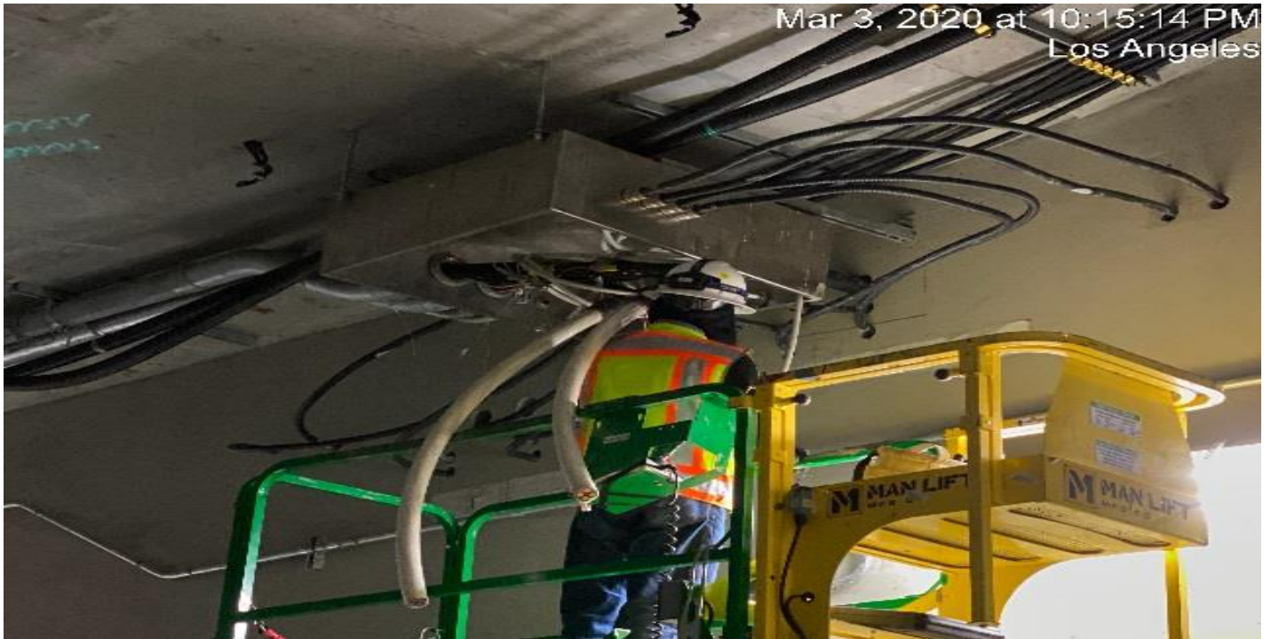
UG4 – Continue wiring and running cable for the booster fans on both north and southbound tunnels at Sta 378+75.
