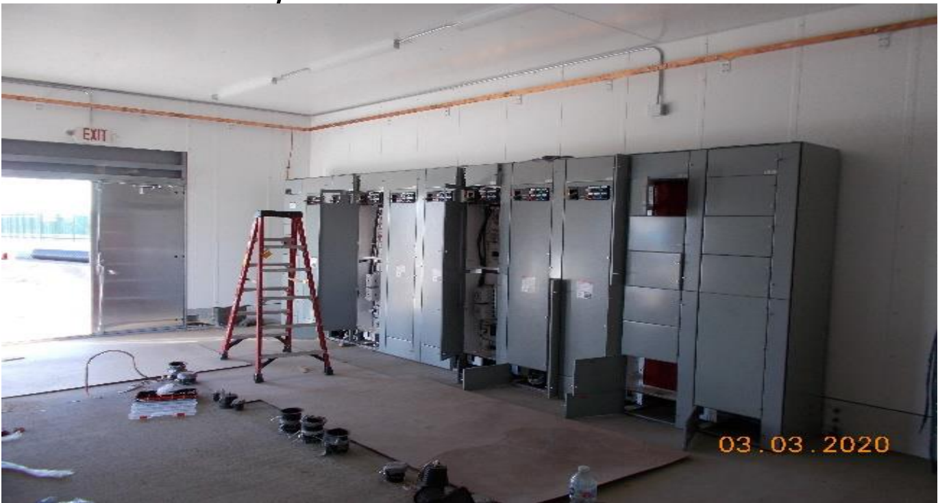
UG3 – Continued placement of MCC sections inside the auxiliary power site bungalow at Victoria Yard adjacent to the south end portal.
