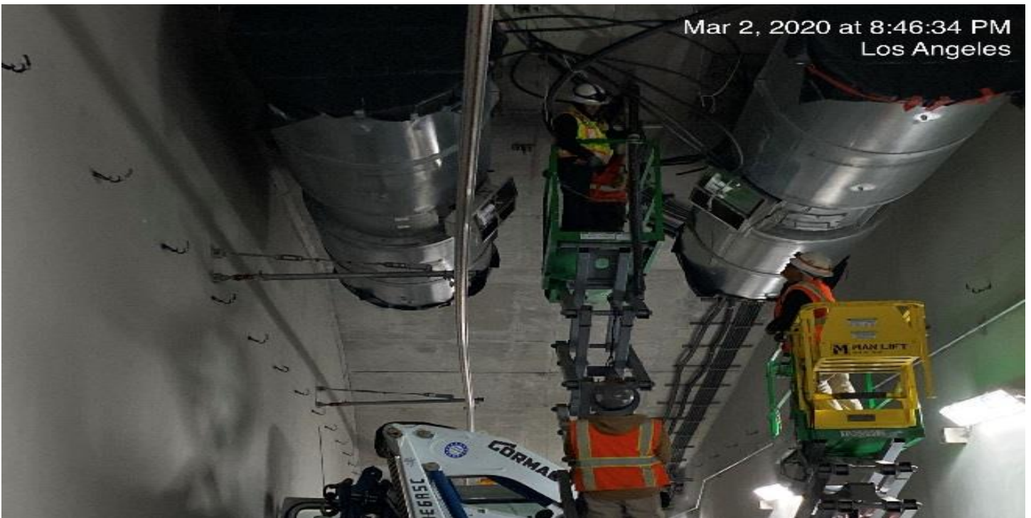
UG4 – Continue wiring and running cable for the booster fans in the northbound tunnel at Sta 378+75.
