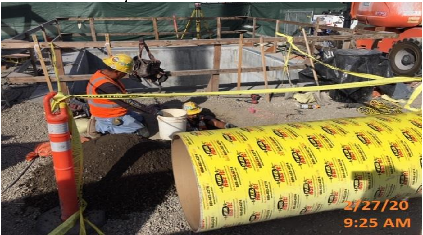
EXPO STATION – Setting sonotube foundation for the installation of the luminaire light posts at the plaza level.
