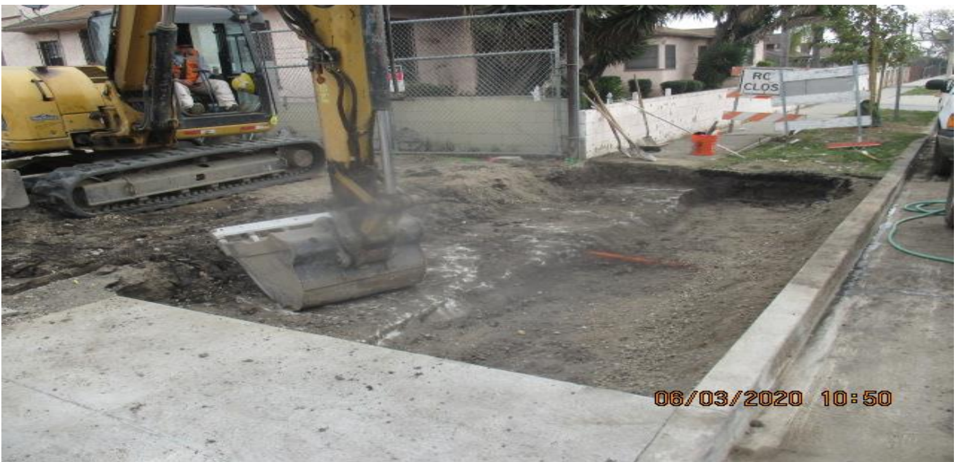
Park Mesa – Excavating for new concrete sidewalk/driveway installation for TPSS#7 entrance on 60th St & Crenshaw Blvd. 3/6/20
