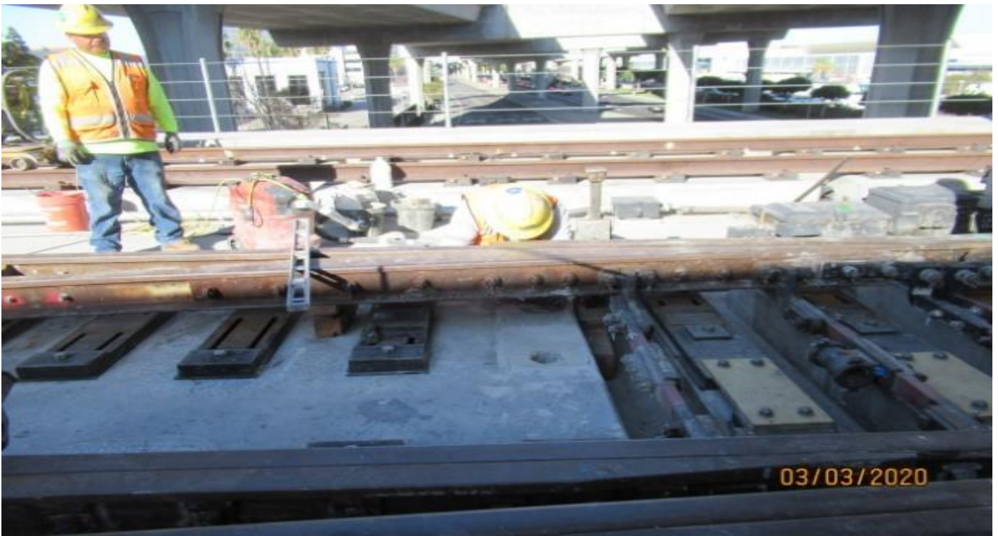
GUIDEWAY - WSCC Concrete foreman hand grinding concrete slab under rails for MPF at GL Wye STA 13+90.
