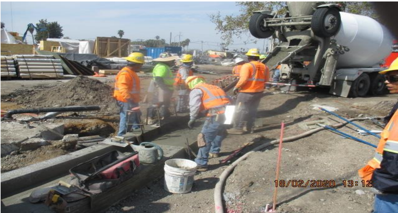
EXPO STATION – Continue curb/gutter formwork and concrete placement for new Cul-de-sac radius sections on Bronson St. east of the plaza. 2/18/20
