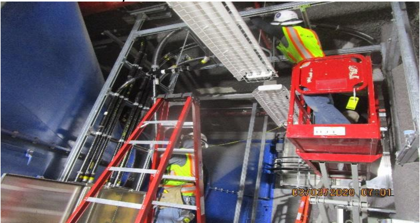
LEIMERT PARK STATION – Continue installing conduit to the pull box for EVF-6-301 in the South Fan Room C – 102 of the concourse level.
