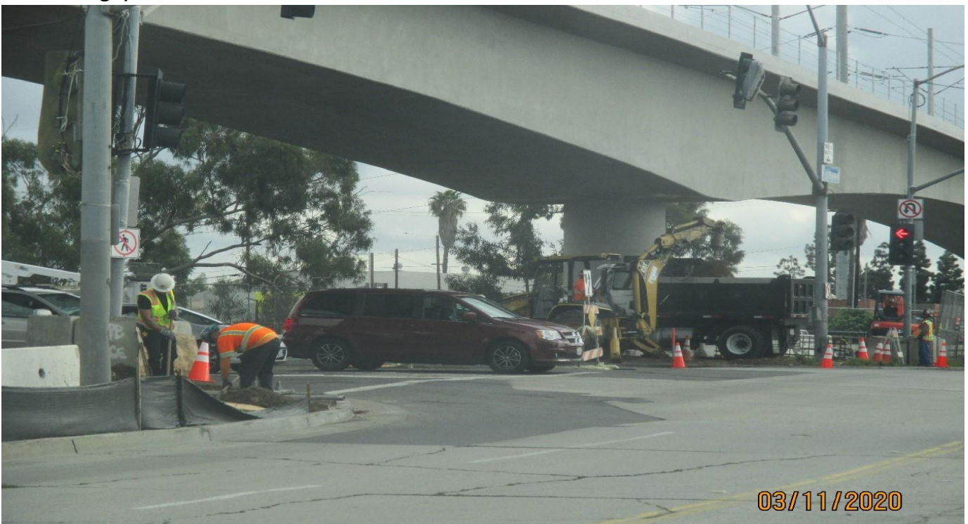
La Cienega/Florence - Excavating for the traffic signal foundations on La Cienega. Facing NE.
