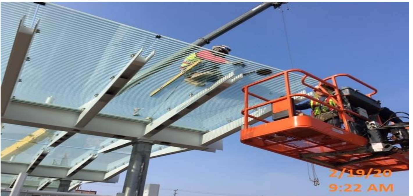
LEIMERT PARK STATION – Continue glass panel installation above the main entrance canopy structure at the plaza level.
