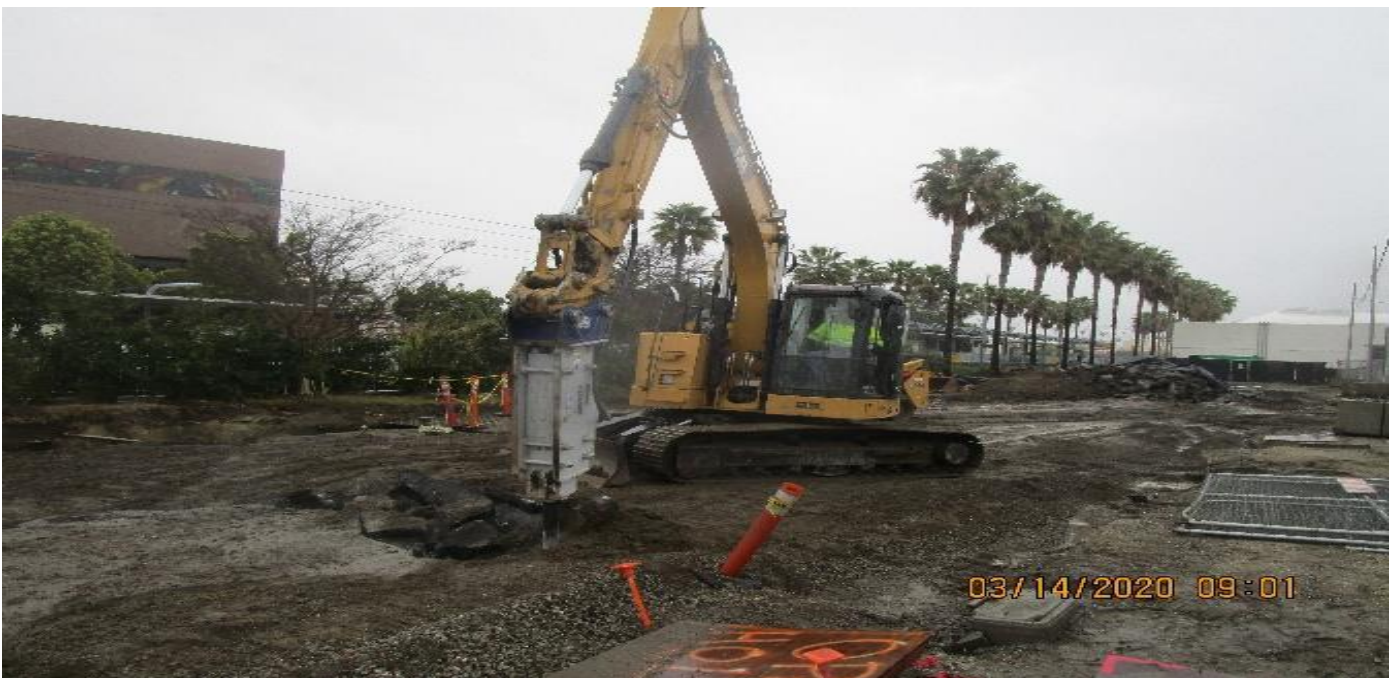
EXPO STATION- Continue demolition/excavation of the roadway east of the plaza in preparation for trenching and underground electrical fiber rough in. 3/14/20.
