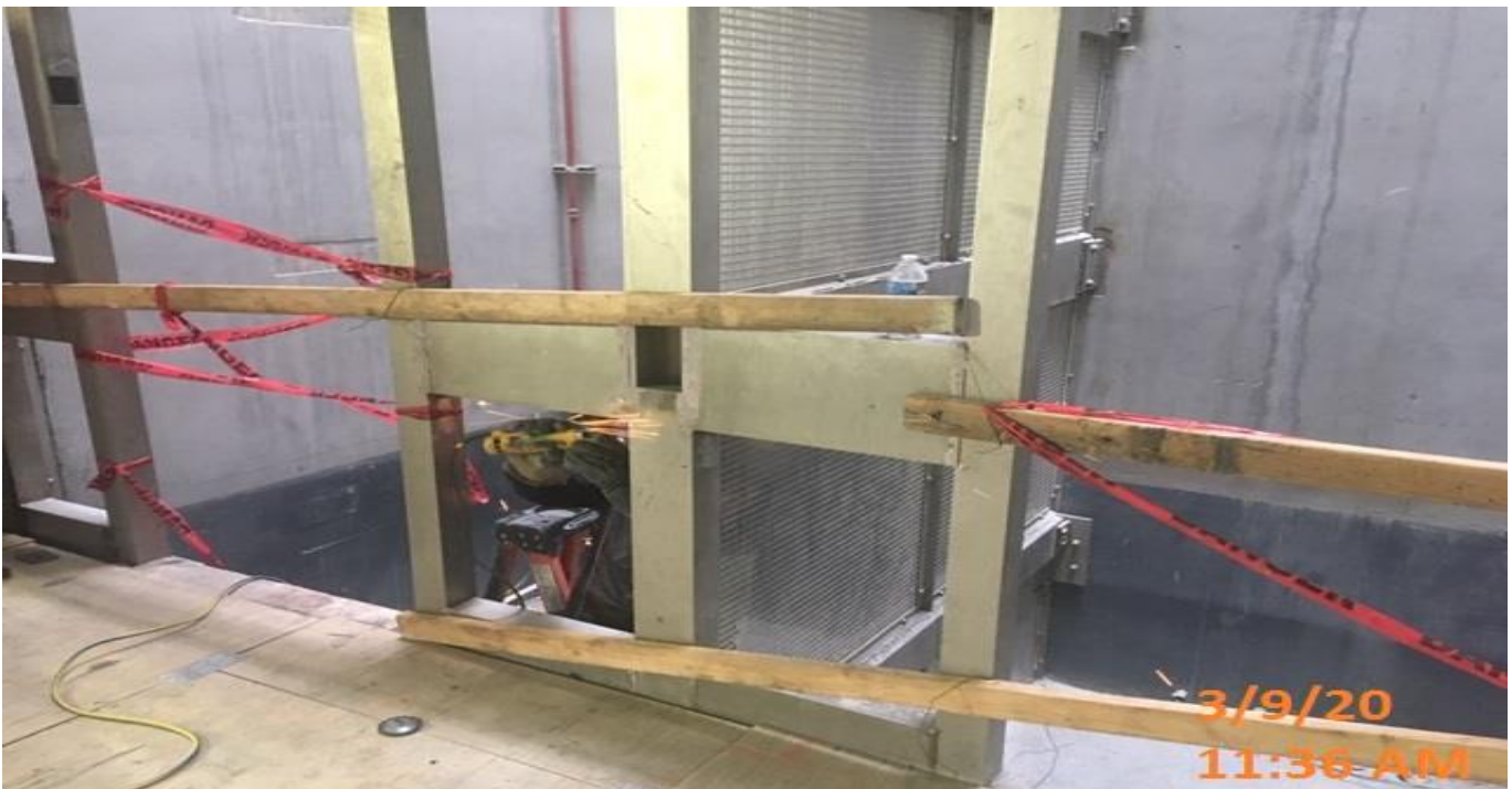
EXPO STATION- Grinding welds on fascia of Elevator Structures 1&2 at the concourse level.
