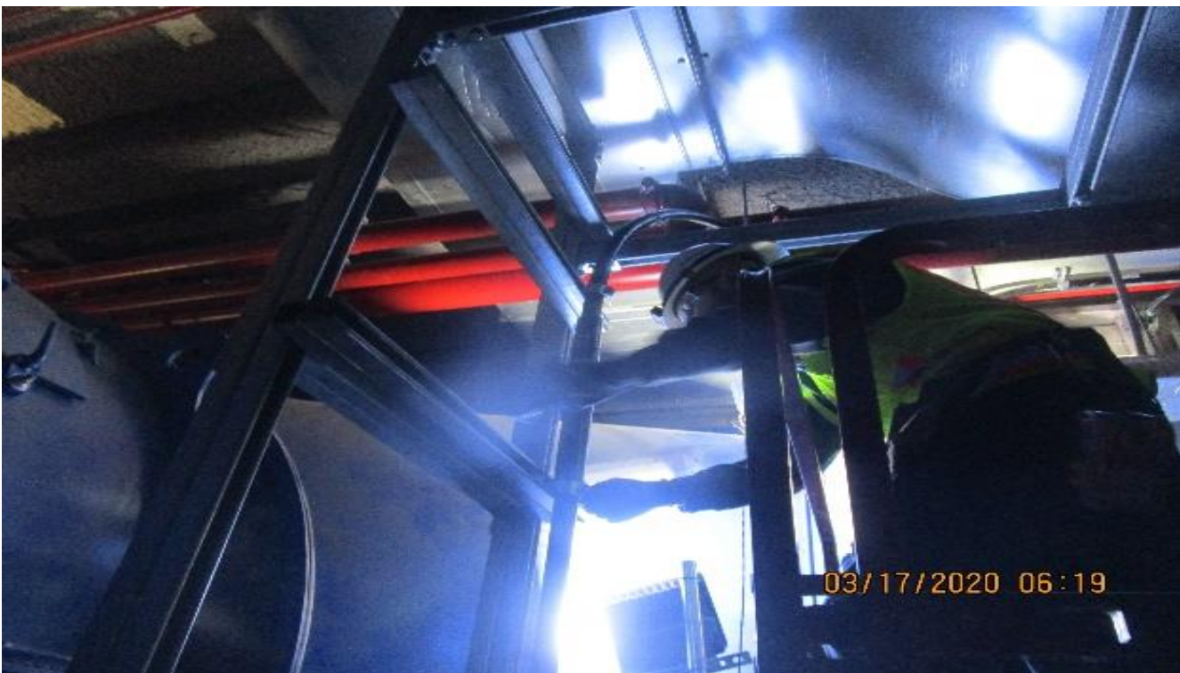
LEIMERT PARK STATION – Continue installing fire rated conduit to the pull box for EVF-6-301 in the South Fan Room C – 102 of the concourse level.
