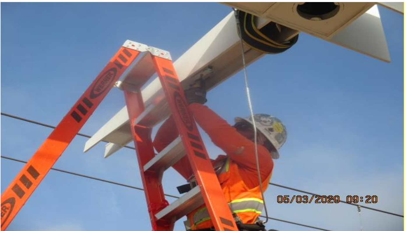
Hyde Park Station – Installing BOCA light fixtures in the out riggers of the canopy roof structure. 3/5/20
