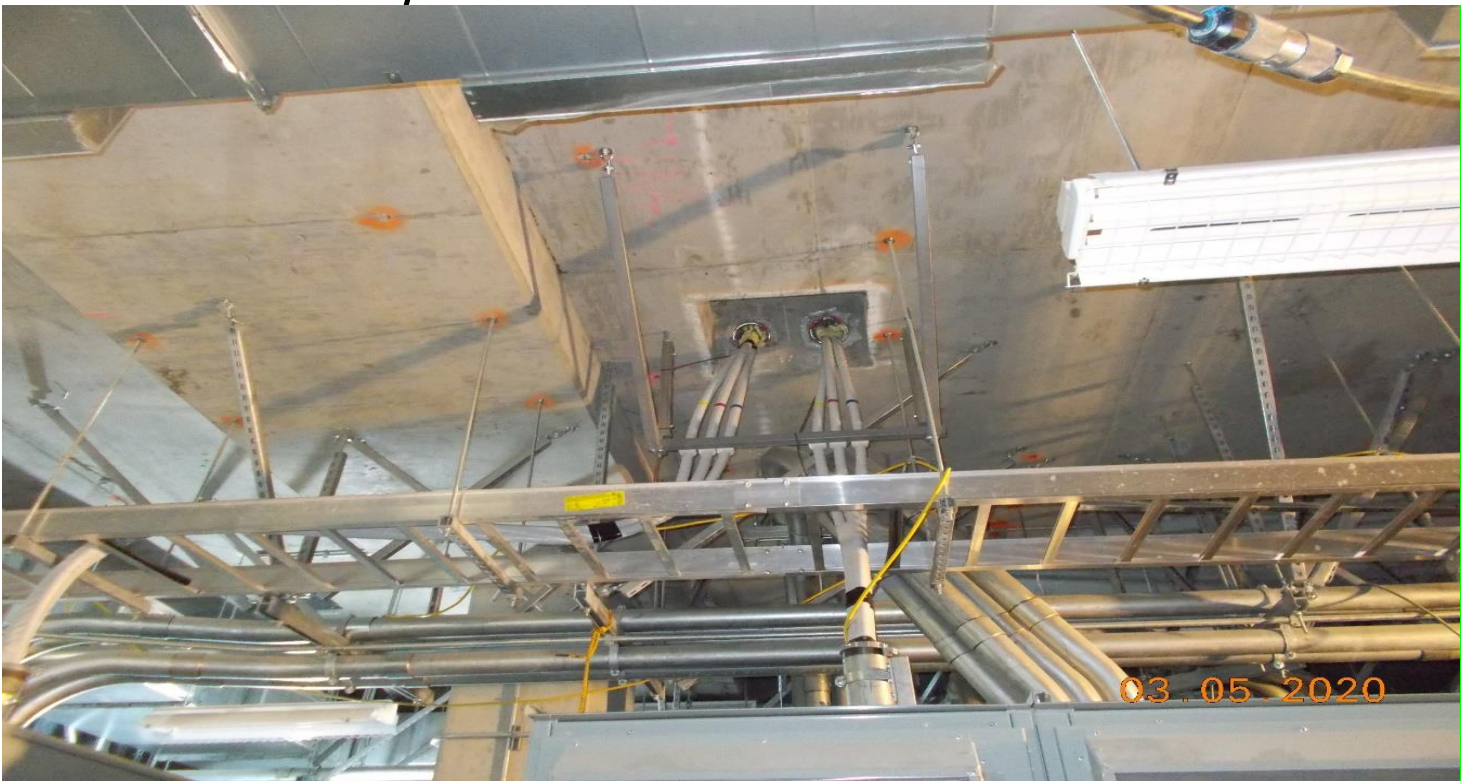
MLK STATION – In Aux Pwr room south Faith Electric had installed a support structure for the high voltage cables.
