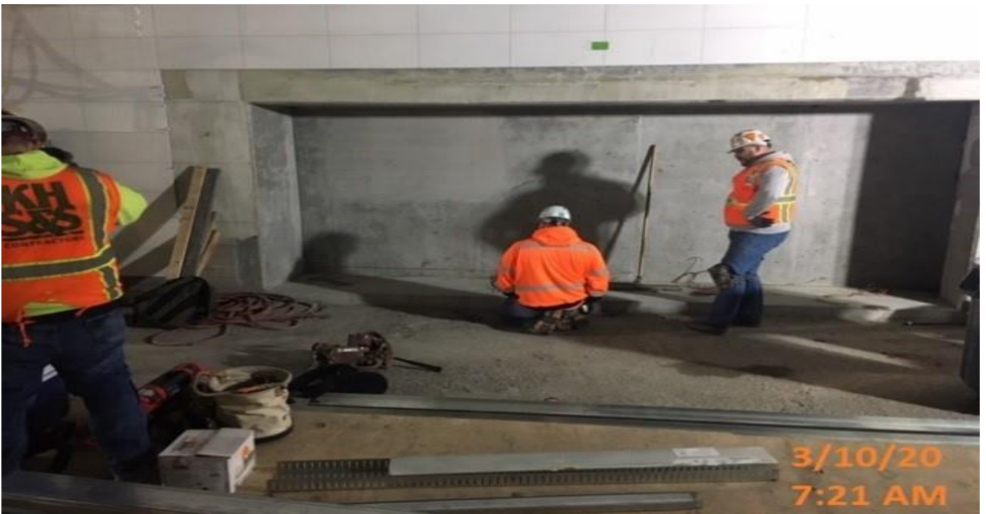
MLK STATION – KHS&S installing steel stud track for ticket vending machine at concourse level.
