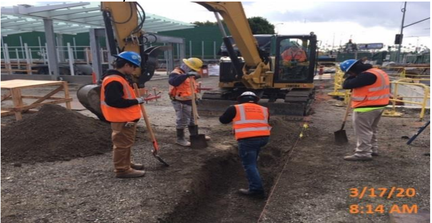
LEIMERT PARK STATION – Excavating trench for the installation of the stainless steel station bollards at the plaza level.
