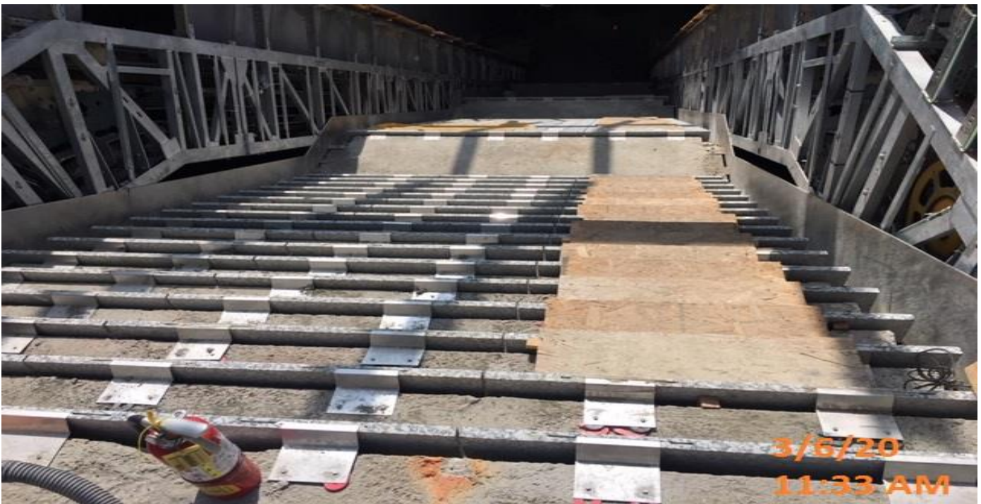
EXPO STATION- Installing granite risers at the main entrance staircase landing of the plaza level.
