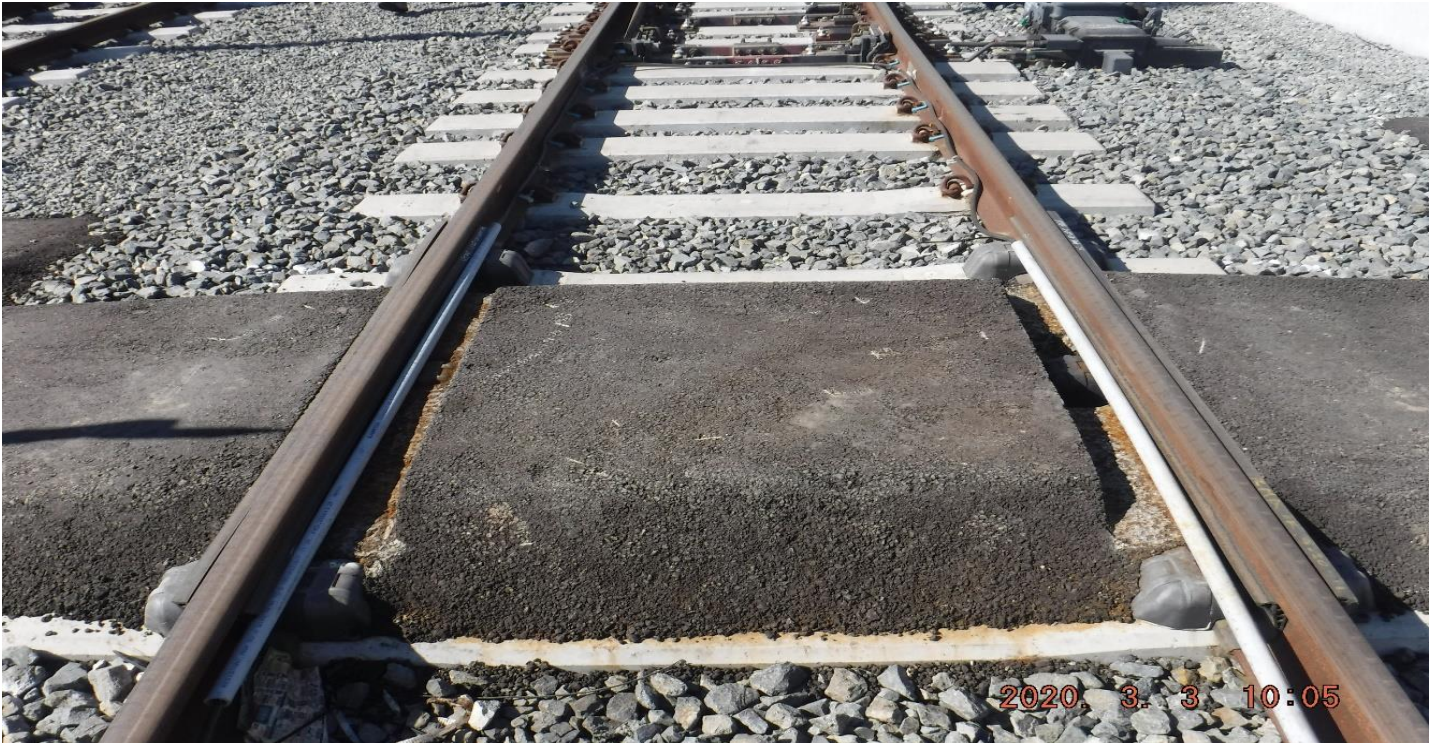
Florence/Ivy - STA255+50_ Looking South_ AC Xwalk before repair between rails_ High
