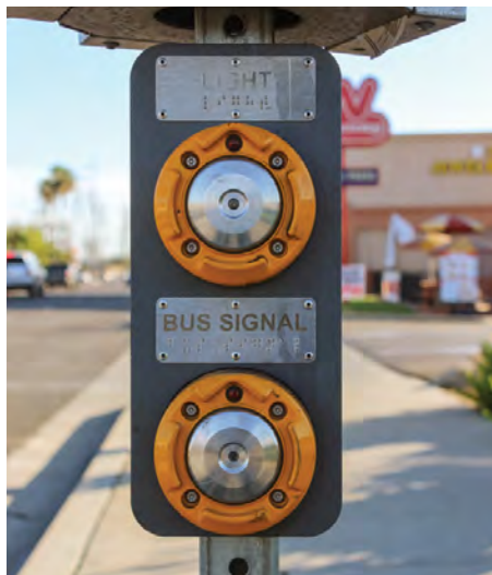
Riders can press a button to activate a flashing light signal for a bus operator to stop. Photo courtesy of Orange County Transit Authority.
