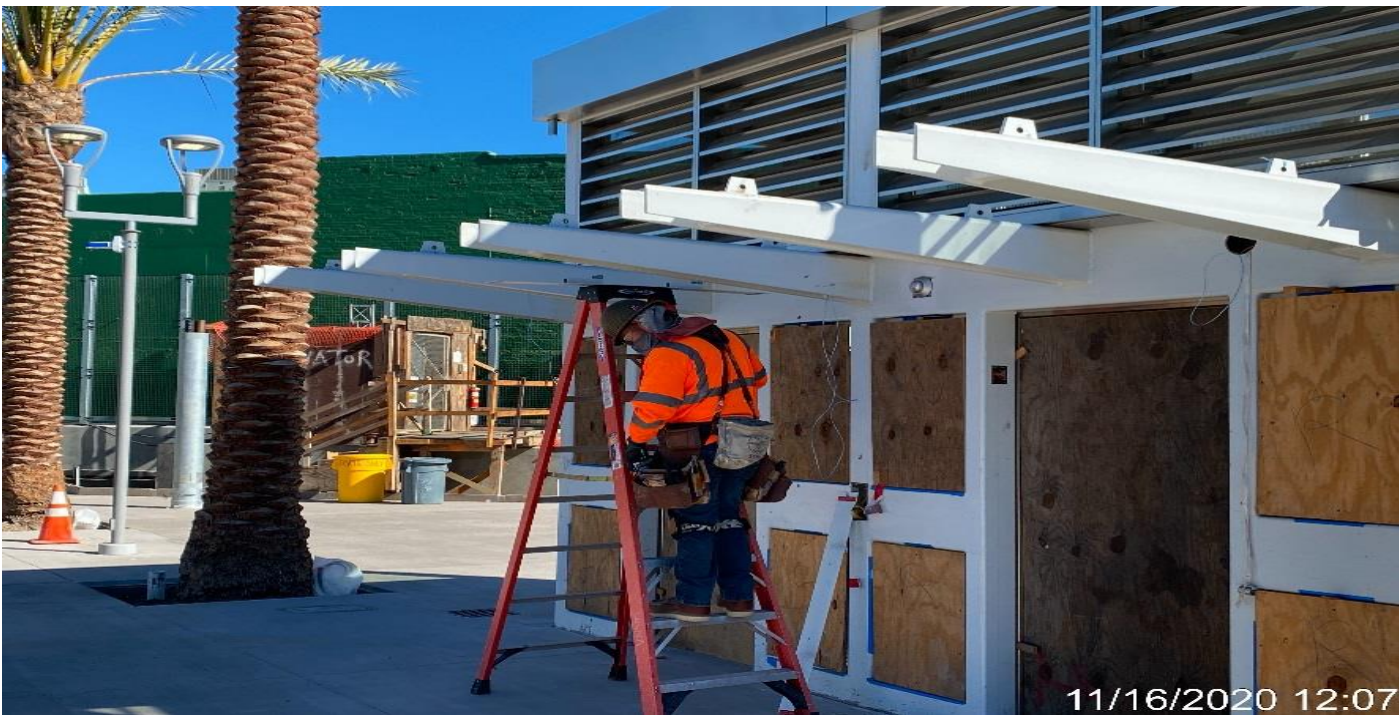
LEIMERT PARK STATION – Installing brackets to canopy outriggers of Elevators 1&2 for BOCA light fixture installation at the plaza.
