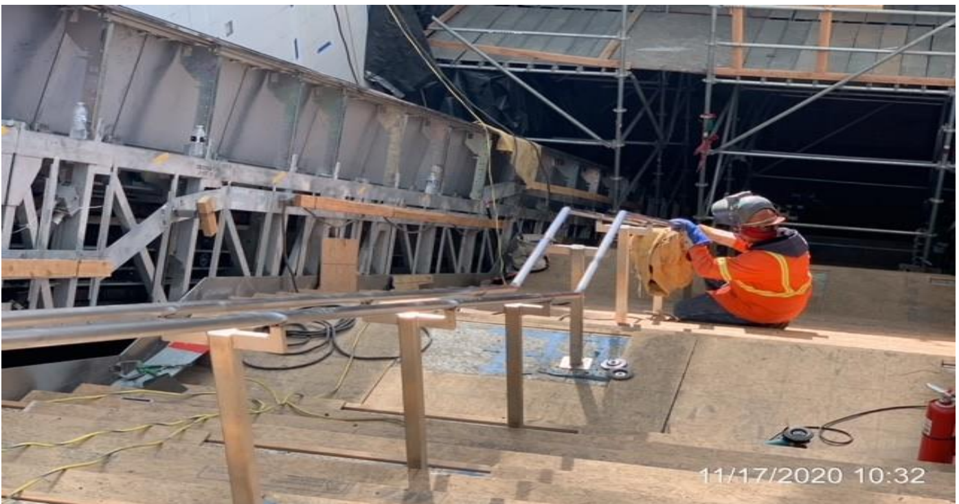
EXPO STATION – Continue installing center handrail for Staircase 1 from plaza to concourse.
