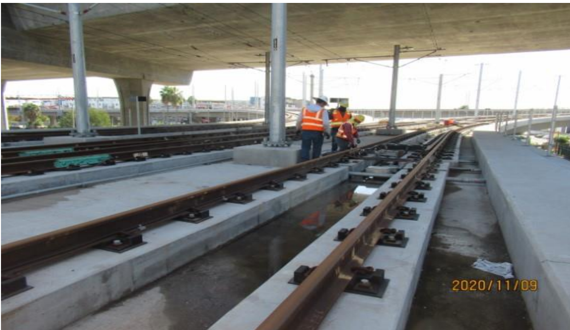
Guideway- WSCC at GL Wye adjusting track gauge on SBW track (looking south) Rework
