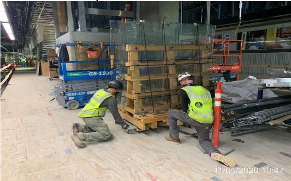
EXPO STATION – Giroux Glass mobilizing glass panels for elevator #3 and #4 at platform.
