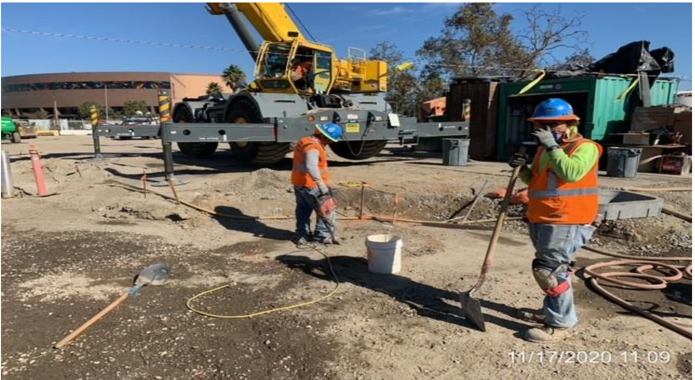
EXPO STATION – Grading and compacting the south end area of the plaza.
