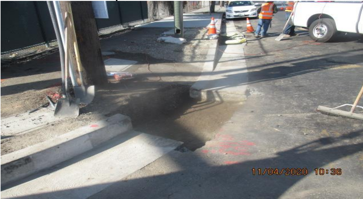
PARK MESA – Saw-cut and excavate for new ADA ramp and curb/gutter installation on the southwest corner of Crenshaw Blvd and 60th St.
