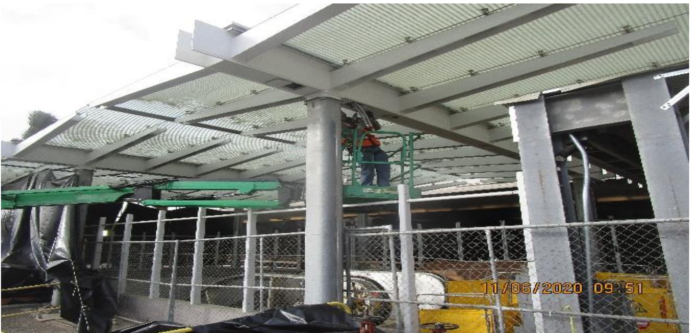
MLK STATION – Continue drilling holes to the main entrance canopy outriggers for BOCA light fixture installation at the plaza.
