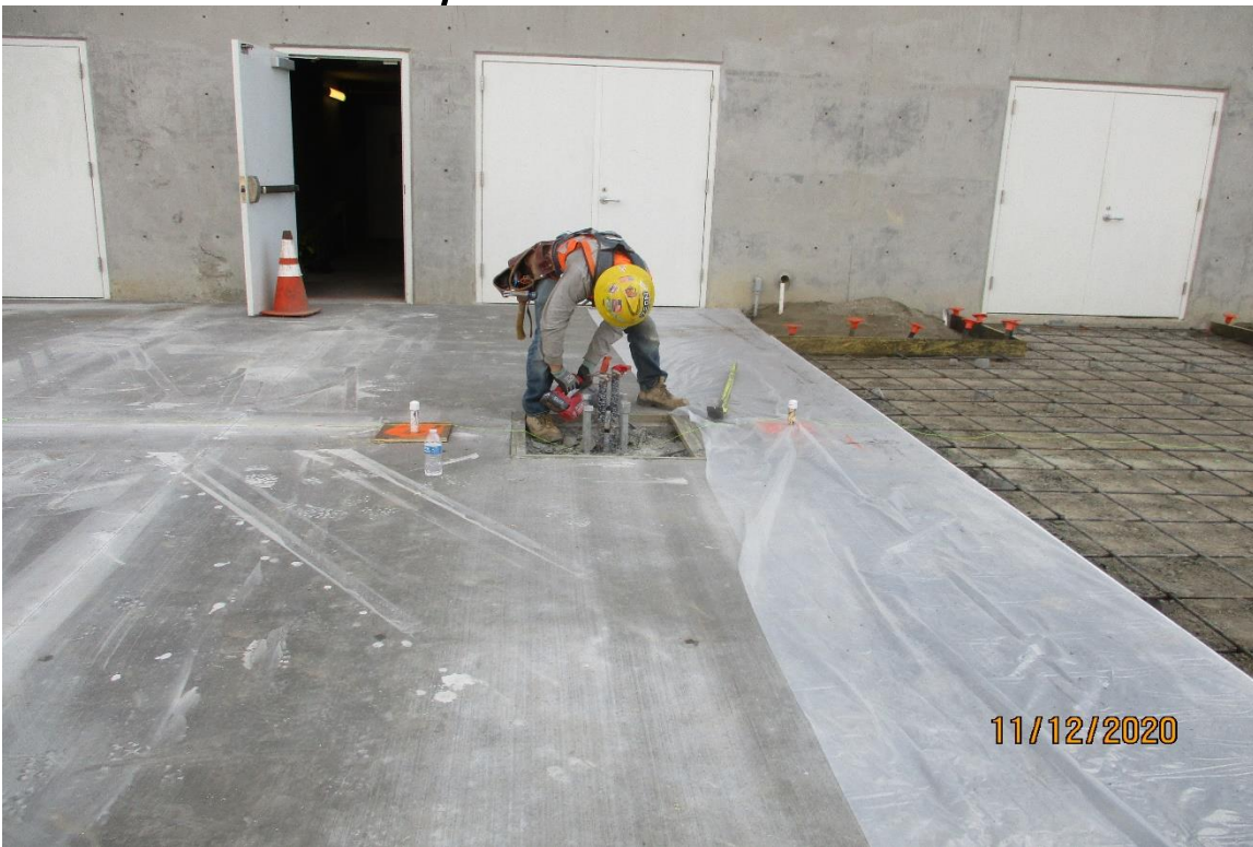
AVIATION/CENTURY- Removing the light pole foundation blockout at the Aviation Station plaza.
