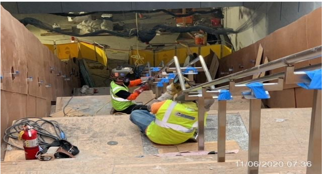
MLK STATION – Continue installing center handrail for Staircase 1 from plaza to concourse.
