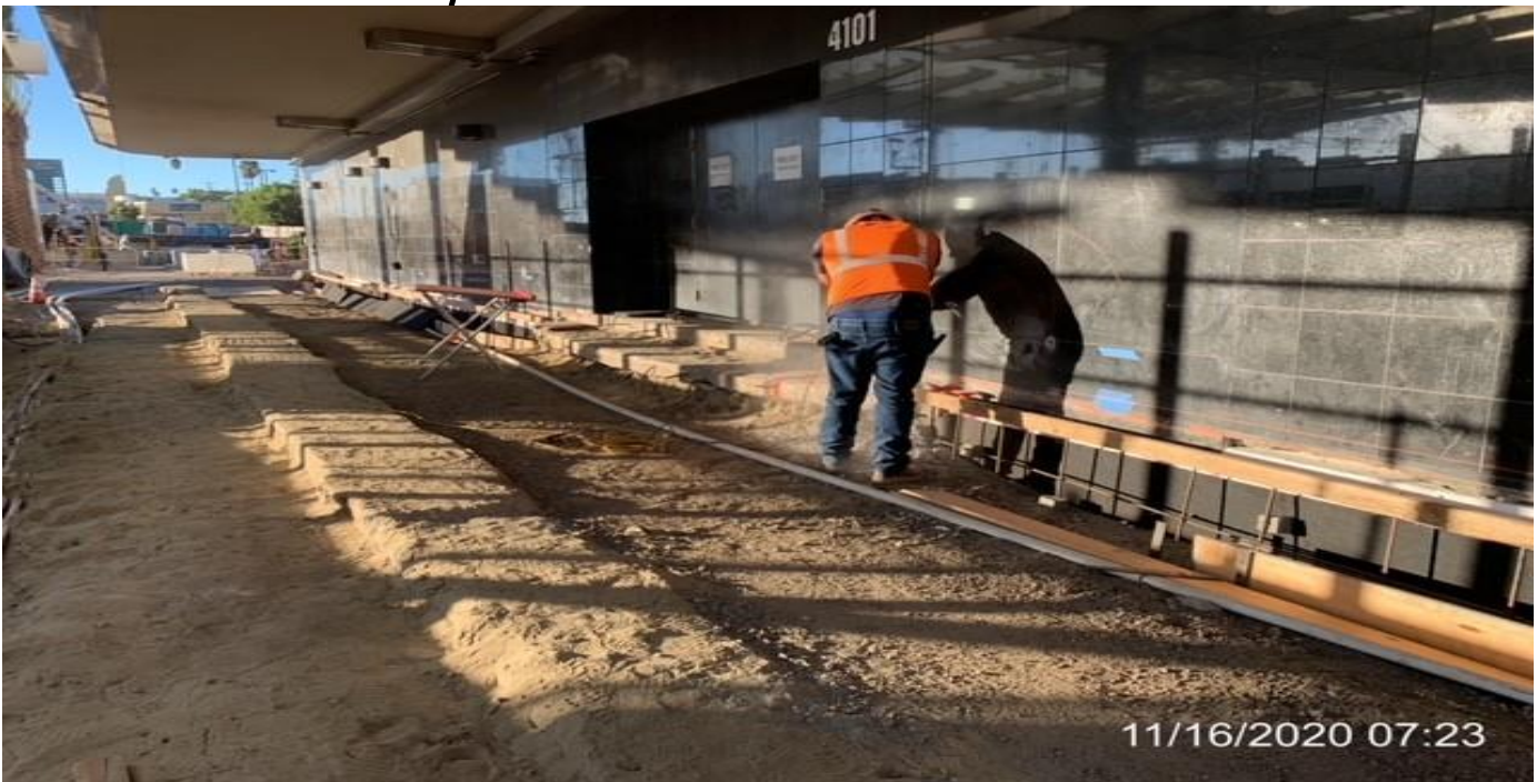
MLK STATION – Chipping door landing of the Mall for curb new walkway curb along the west side of the plaza.
