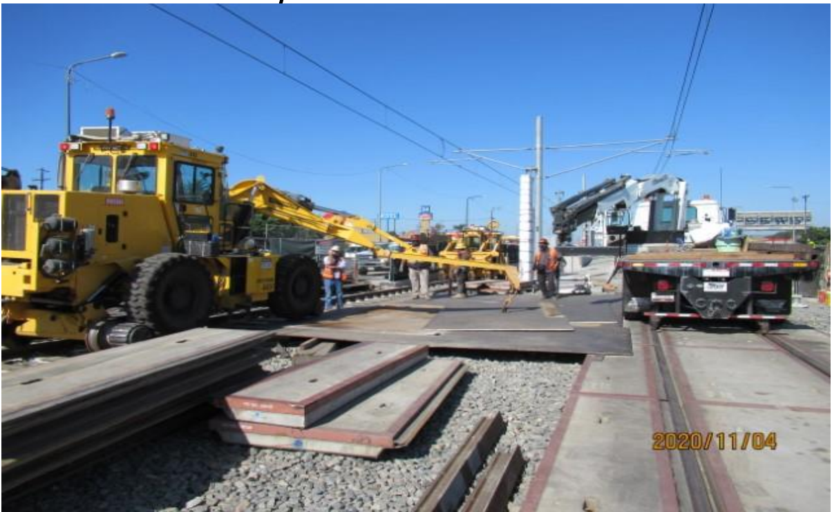
UG3 – WSCC assisting HCC removing shoring plates between tracks using hi-rail Crain truck at 59th Street (looking north) Rework
