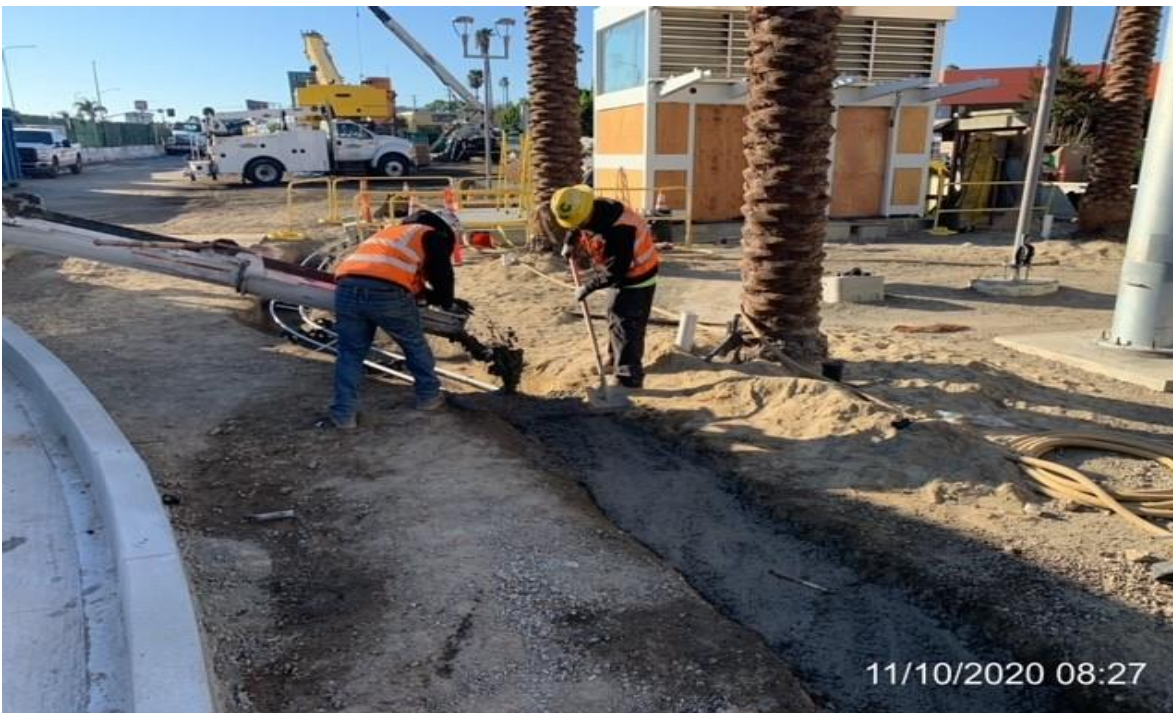
MLK STATION – WSCC crew placing concrete encasement for 1” power and comm conduit.
