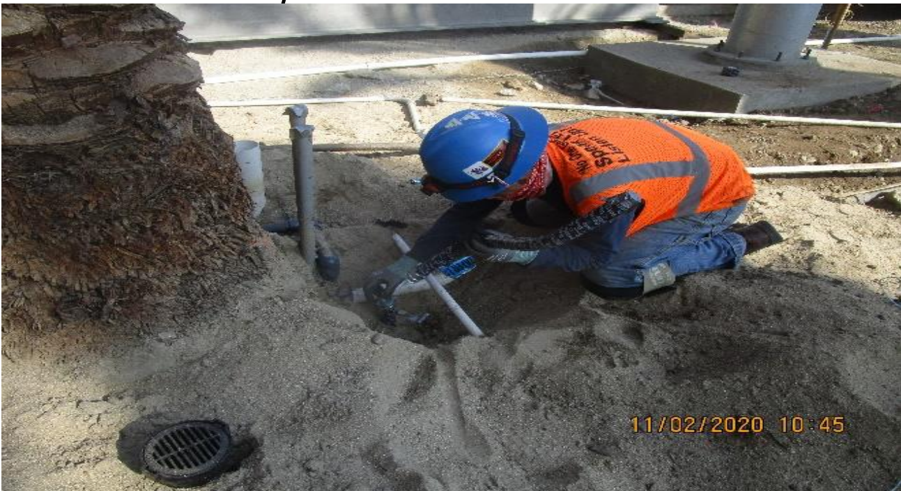
MLK STATION – MLK North Plaza, continued Reworking 1” GRC landscape lighting to allow grate clearance & installation.
