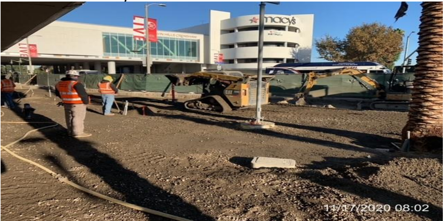
MLK STATION – Continue laying base and compacting the far northwest area of the plaza.
