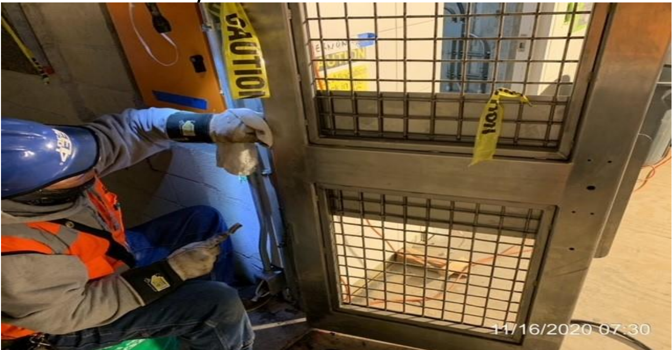
MLK STATION – Grinding and polishing welds for all the platform end gates.
