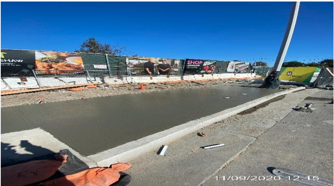
EXPO STATION– Continue placing concrete for sidewalk panels along westbound Obama Blvd and Crenshaw Blvd.
