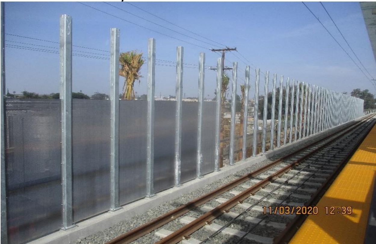
La Brea – ACE Fence Placed special panels on ballast wall at La Brea Sta.
