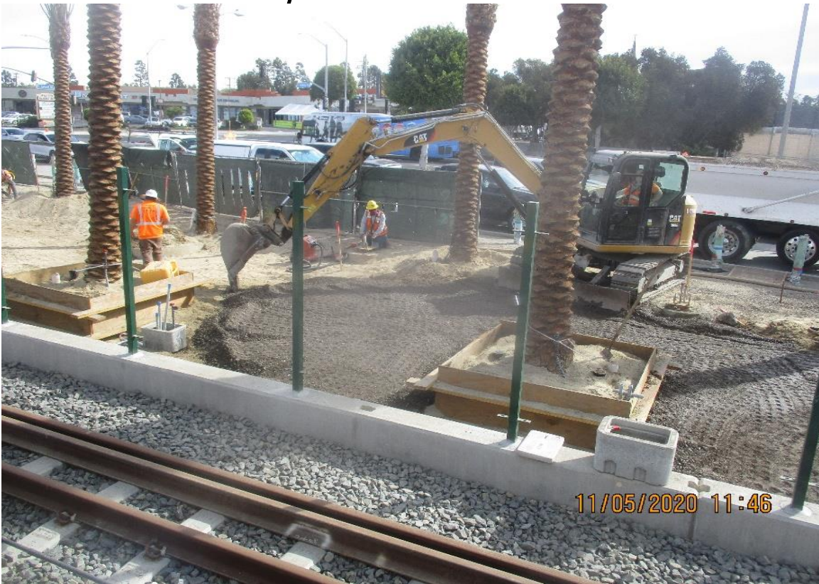
La Brea – Placing concrete for the ADA ramps at the La Brea Station.
