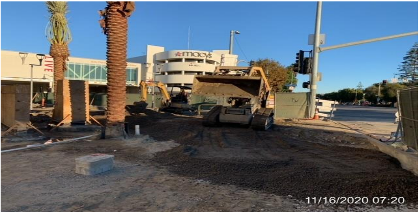
MLK STATION – Laying base and compacting the far northwest and northeast corner area of the plaza.
