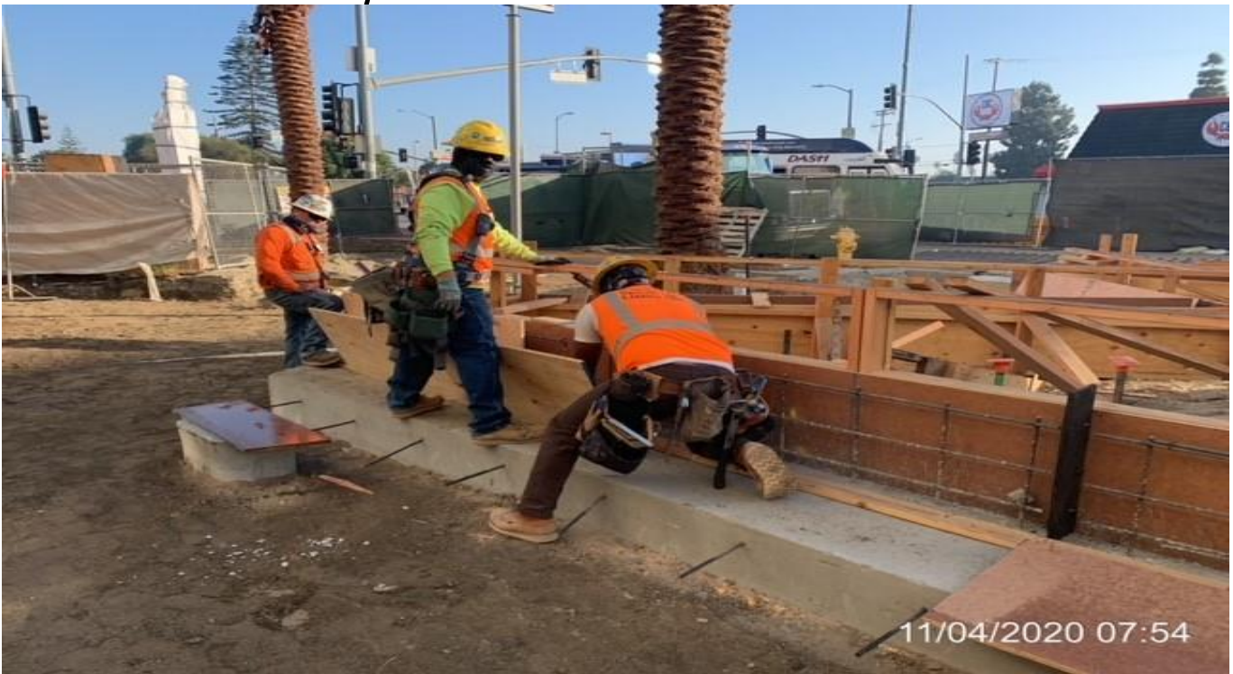
MLK STATION – Continue building formwork for the north planter wall at the plaza.
