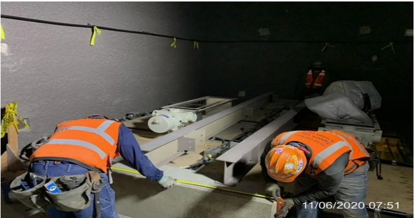
MLK STATION – Anchoring steel I-beams for catwalk installation in the Tunnel Vent/OTE Plenum North C-143 at the concourse.
