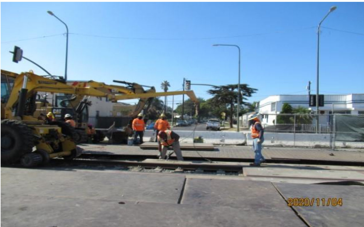
UG3 – HCC/WSCC at 59th Street removing crossing panels on SB track for re-tamping through crossing (looking west) Rework
