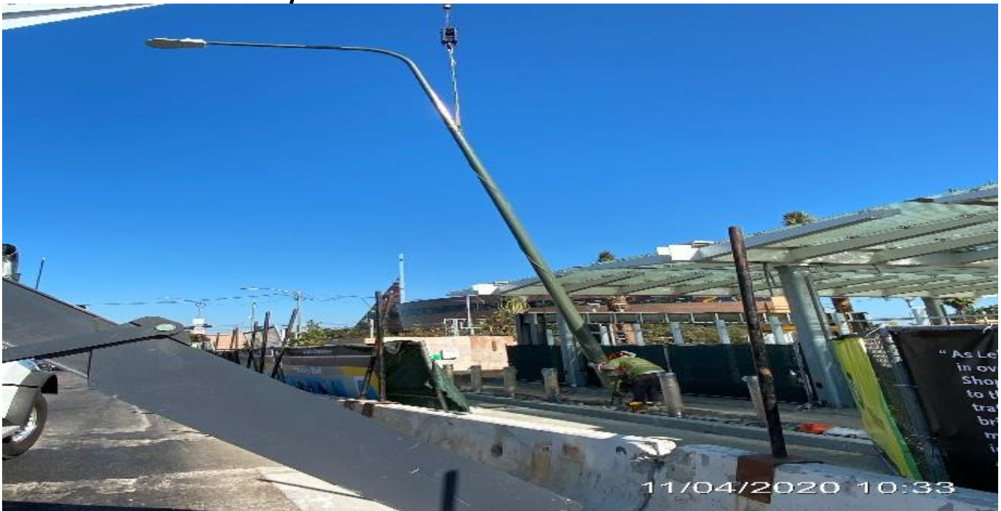
EXPO STATION SITE – Placing pedestrian light poles along the west side of the plaza.
