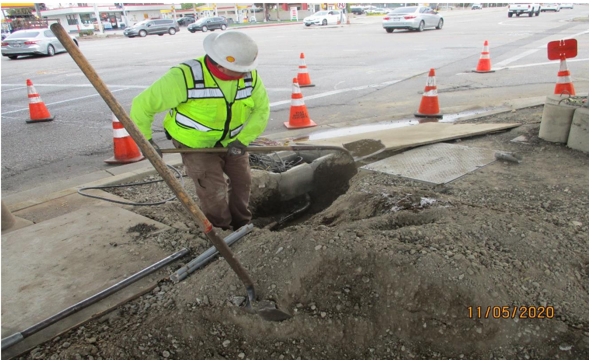
AVIATION/CENTURY- Exposing traffic signal conduit to find a kink in the line on Aviation and Century.
