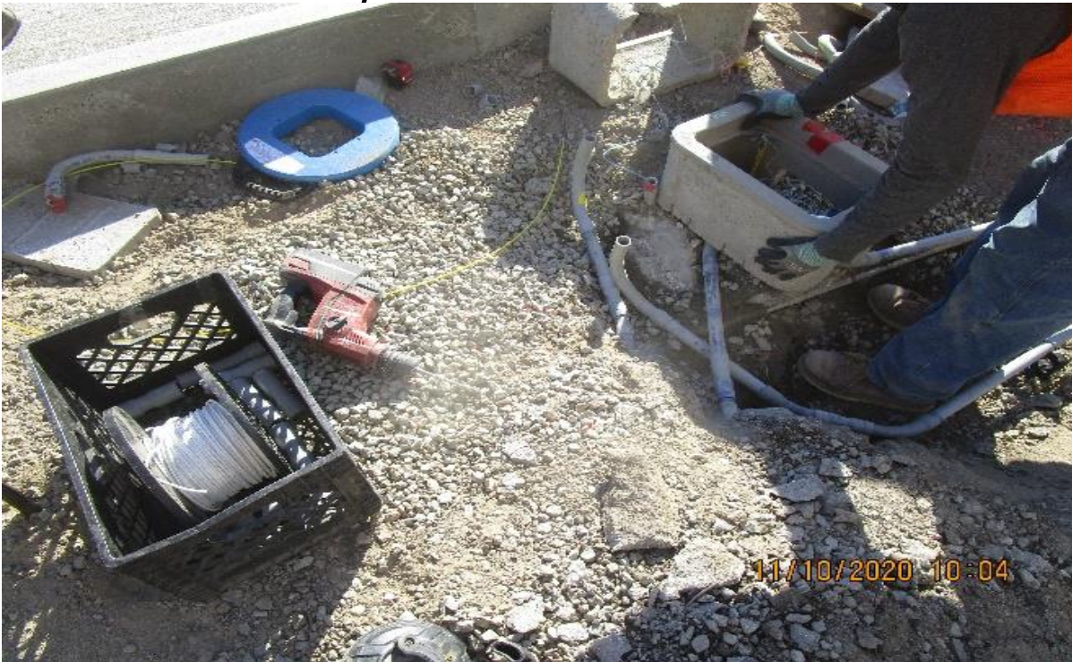
MLK STATION – MLK South Plaza, continued rework of CCTV PVC conduit & setting embedded pull box to elevation.
