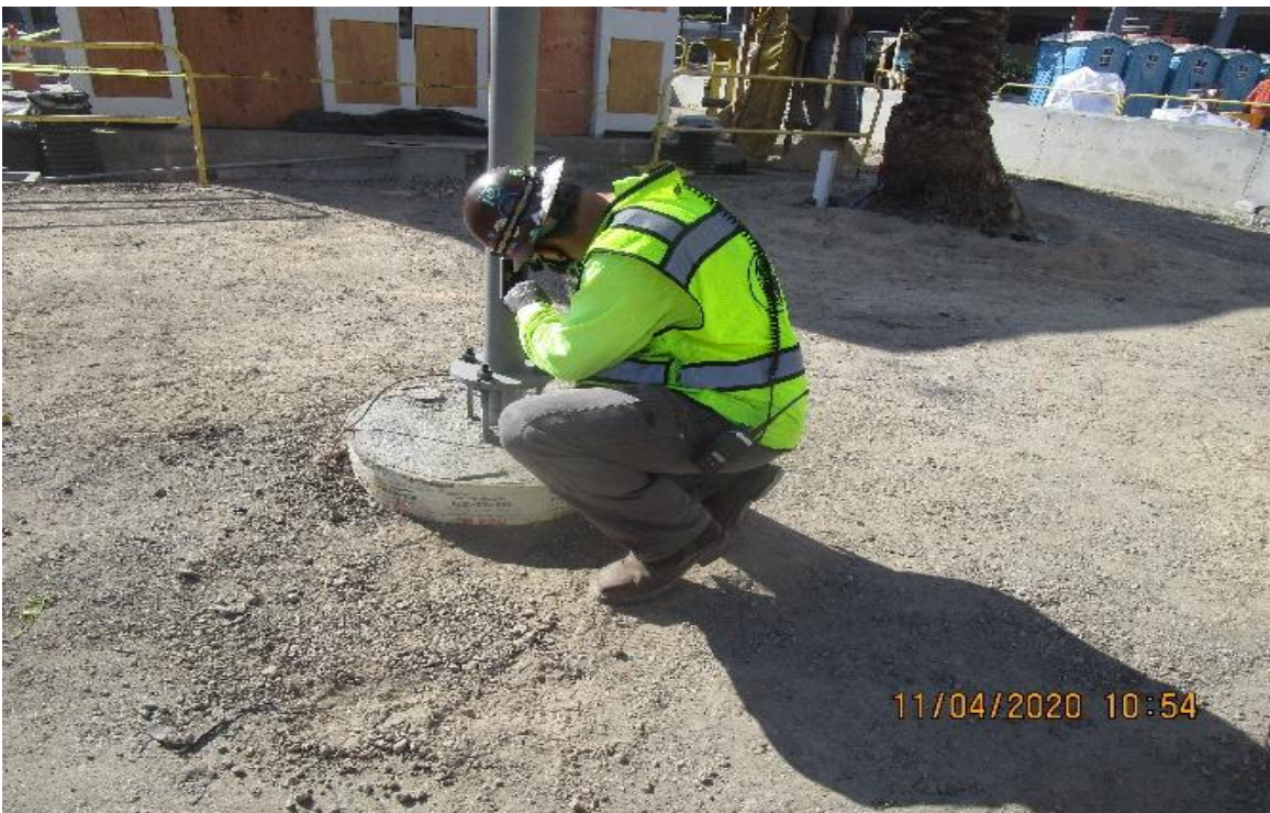
MLK STATION – MLK South Plaza, begin taking measurements for CAT-6 cables at light standards for CCTV cameras.
