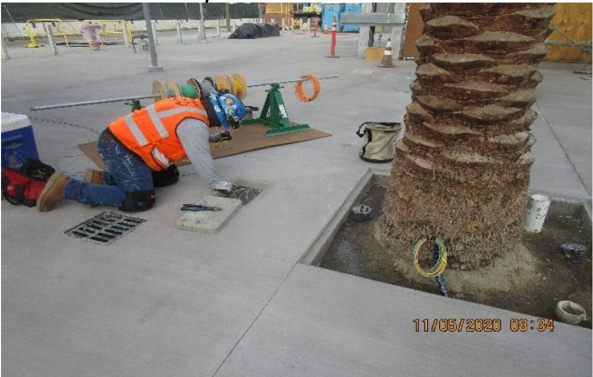
Leimert Park – Vernon Plaza, continued pulling #10 HHW-2 wiring landscape lighting load conductors & grounds.
