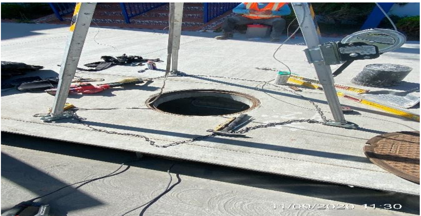
LEIMERT PARK STATION – Sacking and patching CB#1 on SB Crenshaw Blvd between Vernon Ave and 43rd Pl.
