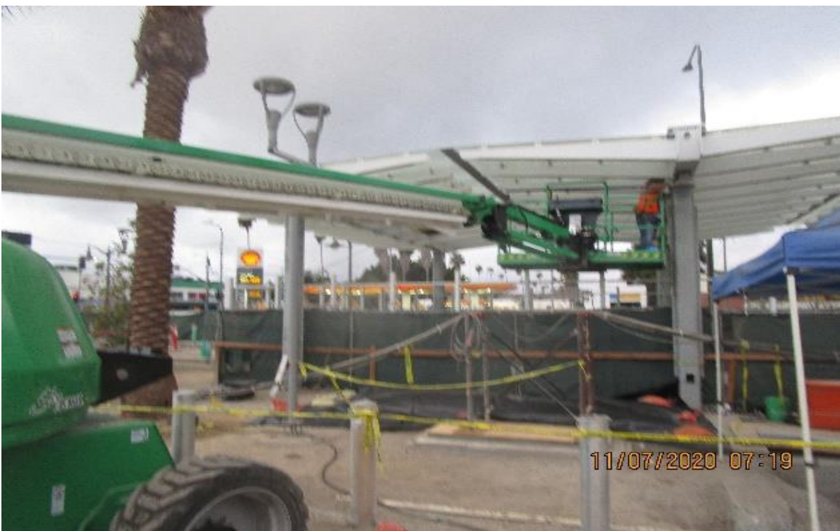
EXPO STATION – Entrance canopy, continued rough in 4' & 8' BOCA LED normal & emergency lighting fixtures.
