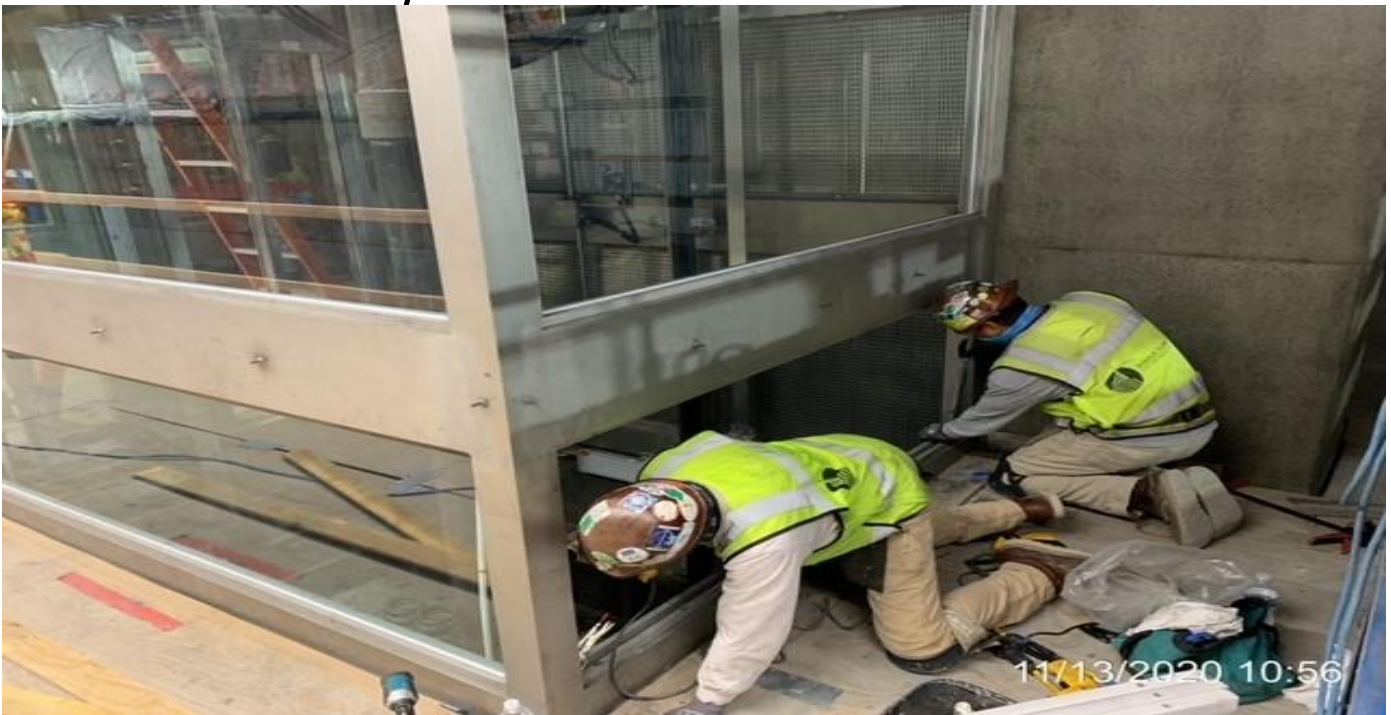
EXPO STATION – Continue installing glass stops and panels to Elevators 3&4 at the platform.
