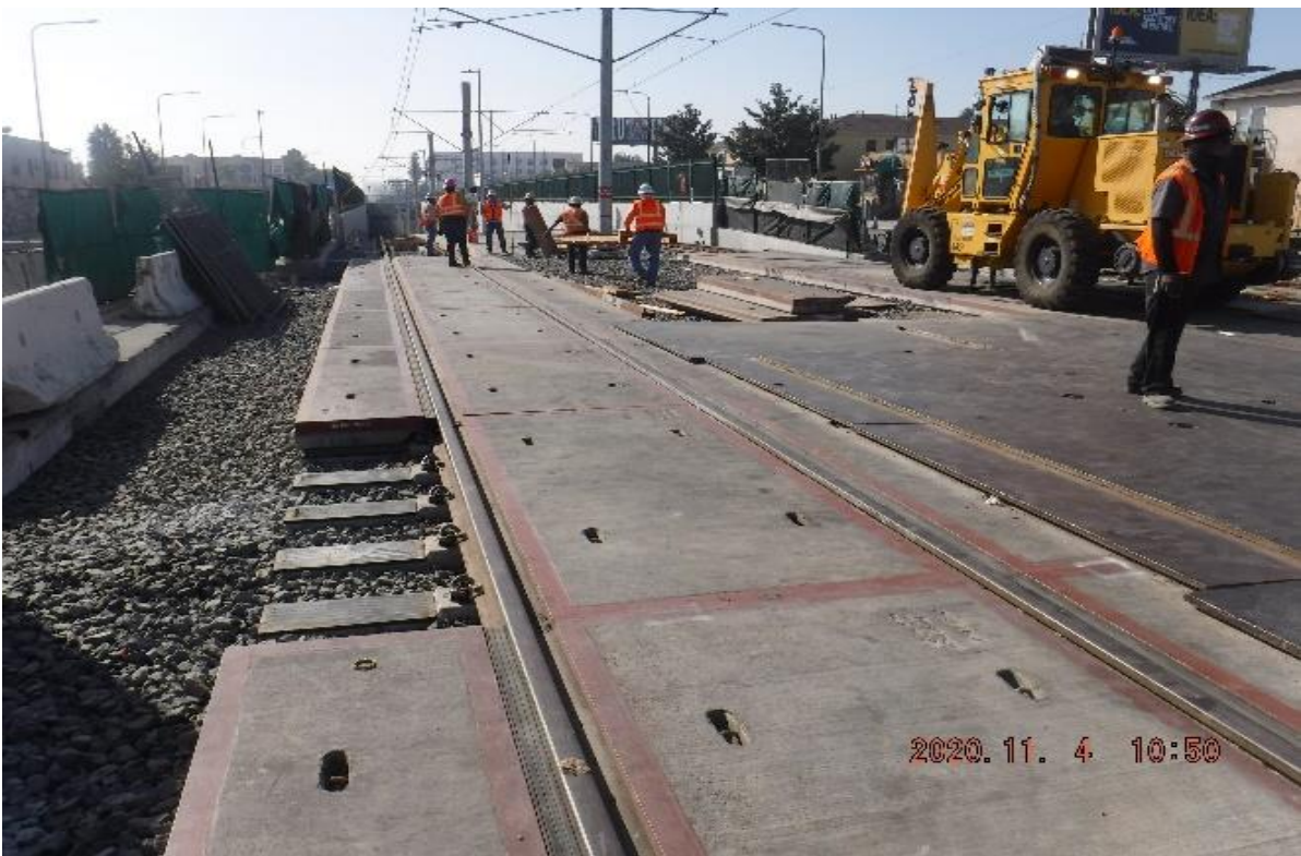
UG3 – STA 317+00 TK#4/NB looking south – 59th St at grade crossing work by WSCC and HCC started.
