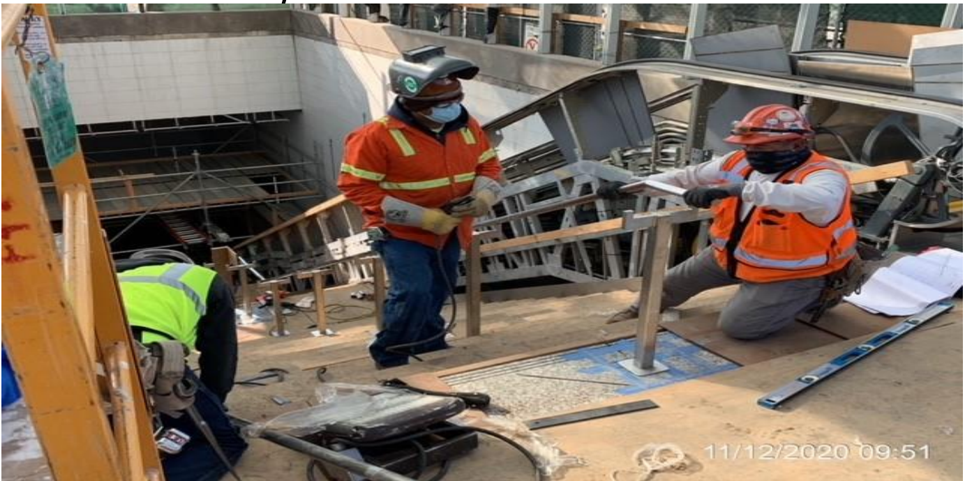
EXPO STATION – Continue installing center handrail for Staircase 1 from plaza to concourse.
