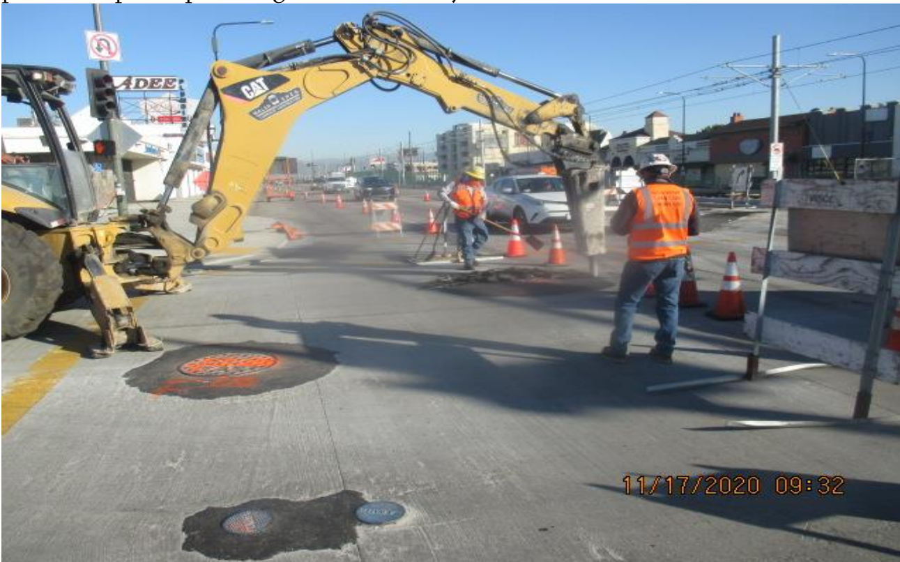
PARK MESA – Removing rings and access covers of sewer maintenance holes in preparation for grind and overlay of southbound Crenshaw Blvd and 57th St.
