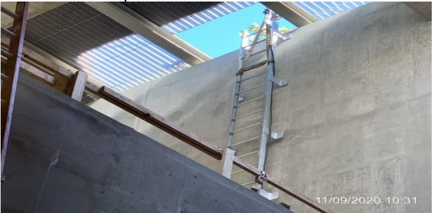
EXPO STATION – Installing steel ladder inside the North Emergency Ventilation Shaft from plaza to concourse level.
