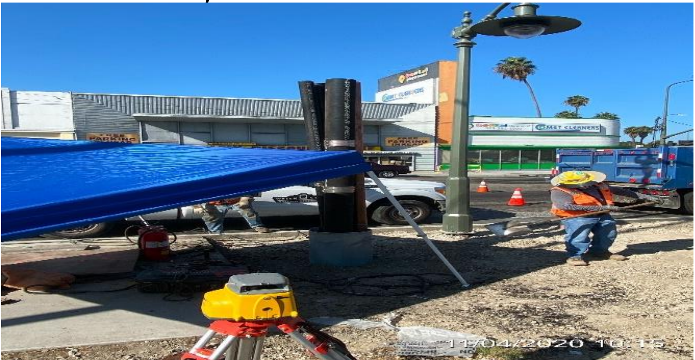
EXPO STATION– Welding stainless steel encasement onto the South Vent Sack base on NB Crenshaw Blvd and Obama Blvd.
