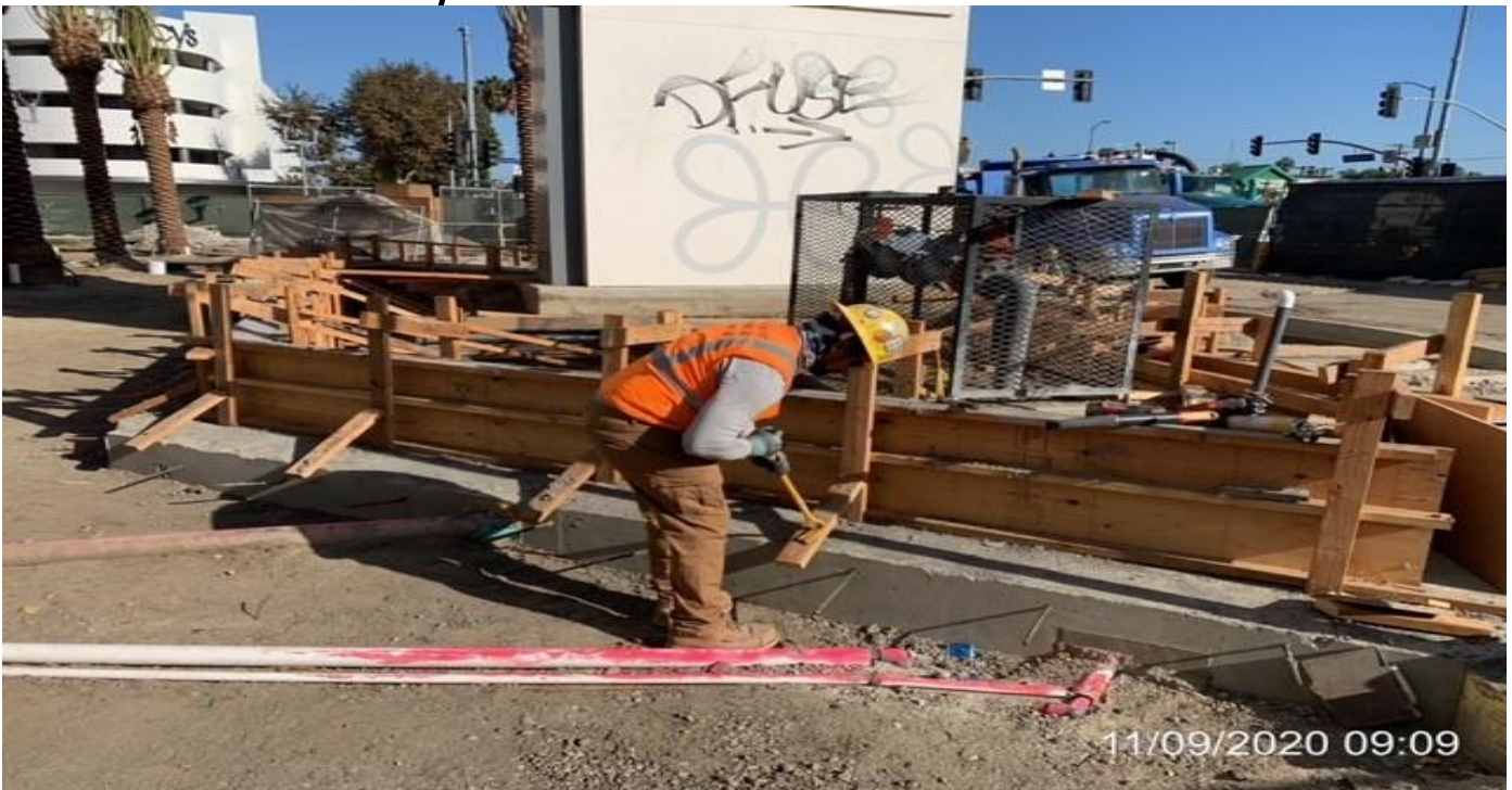
MLK STATION – Continue building formwork for the north planter wall at the plaza.
