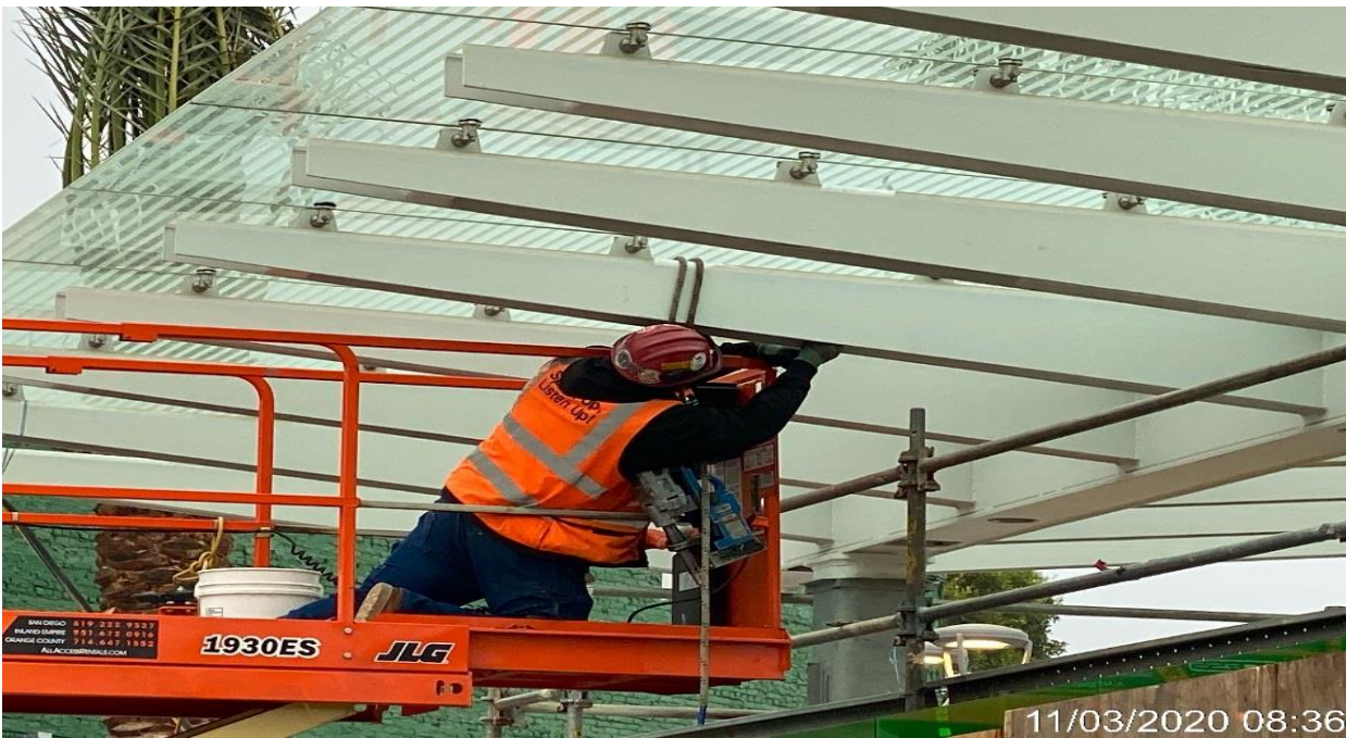
LEIMERT PARK STATION – Drilling holes to the main entrance canopy outriggers for BOCA light fixture installation at the plaza.
