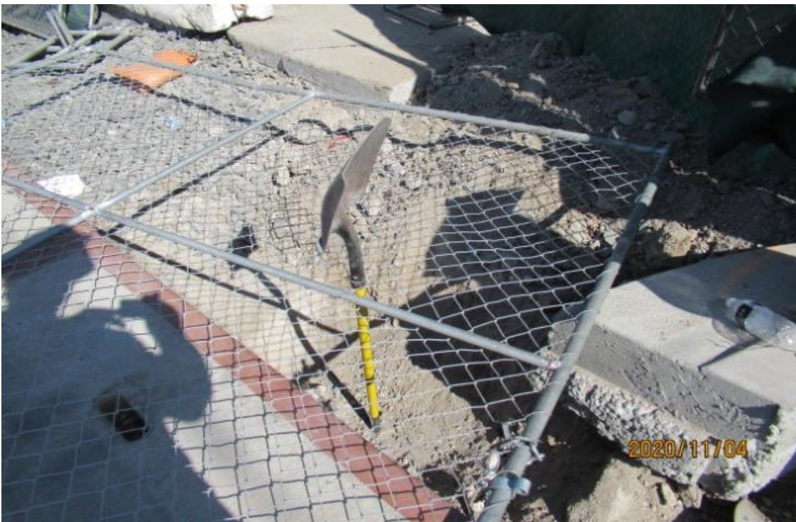
UG3 – 59th Street NB track southeast corner sub-grade compromised to be repaired Rework.
