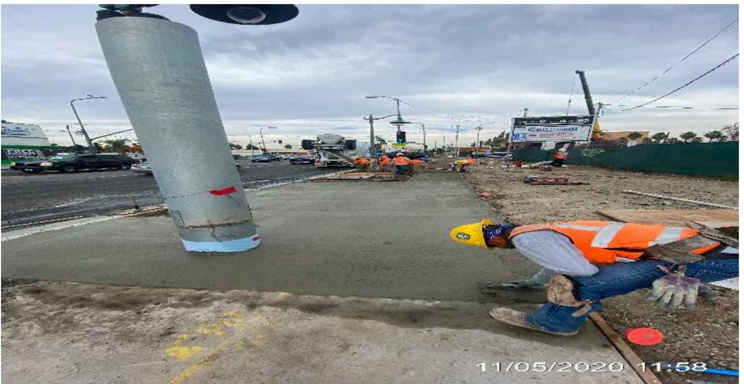
EXPO STATION – Continue placing concrete for sidewalk panels along westbound Obama Blvd and Crenshaw Blvd.
