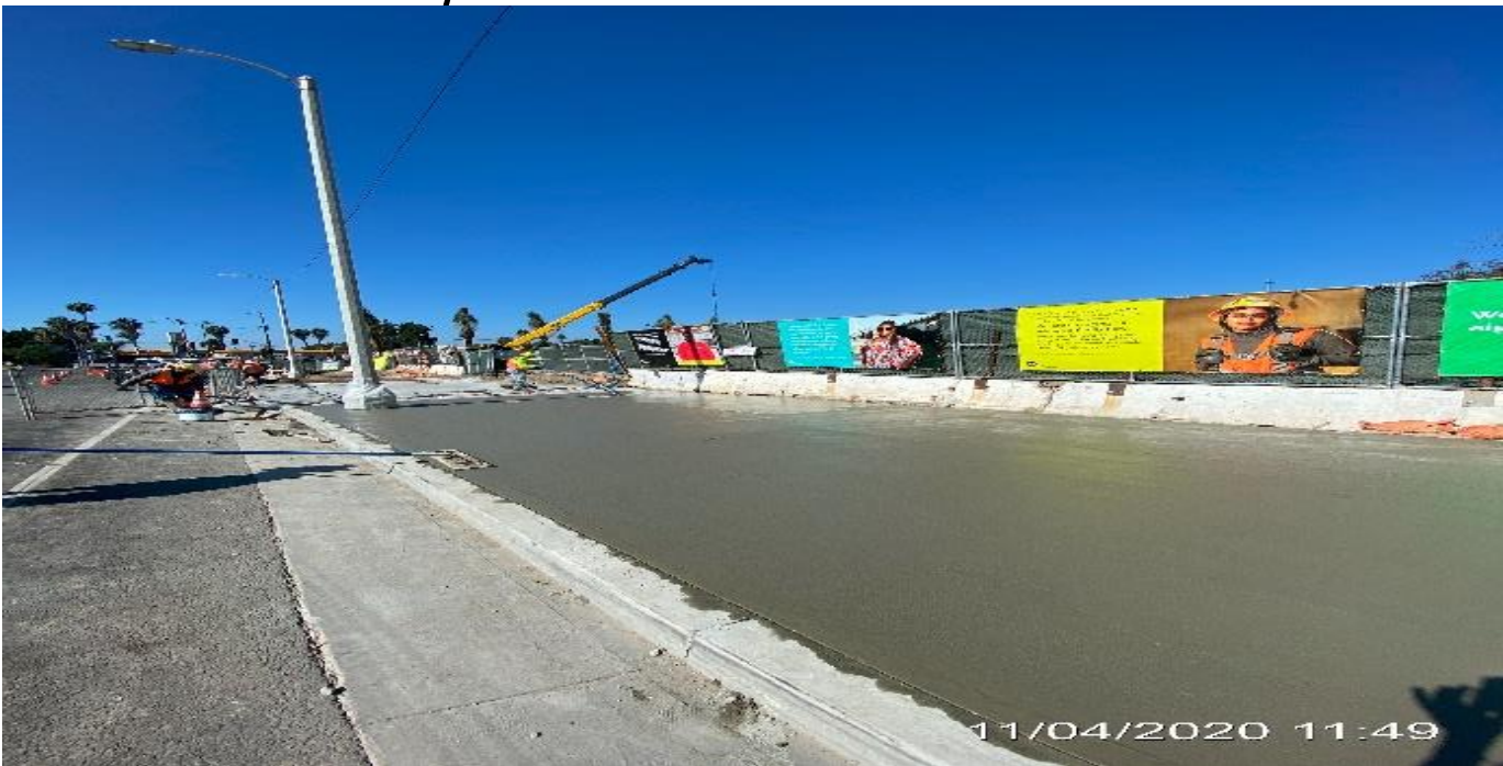
EXPO STATION – Built formwork and placing concrete for sidewalk panels along westbound Obama Blvd and Crenshaw Blvd.
