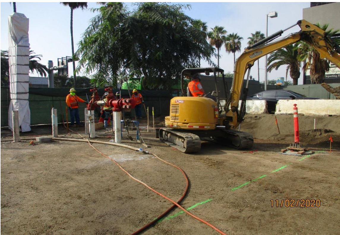
AVIATION/CENTURY- Fine grading the base subgrade at the Aviation Station. Facing SW
