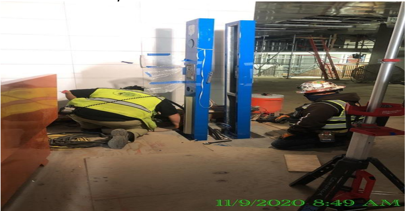
EXPO STATION – Drilling and anchoring free standing GTEs at the Paid Area of the concourse.
