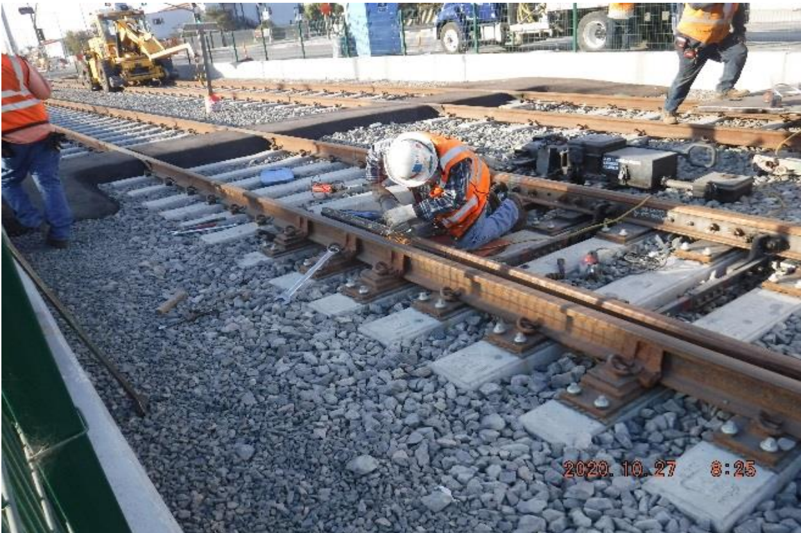
57 th Street – STA 332+53 TK#4/NB looking south – finishing custom manganese insert replacement of 10U1LHXO (divert) (57th St)
