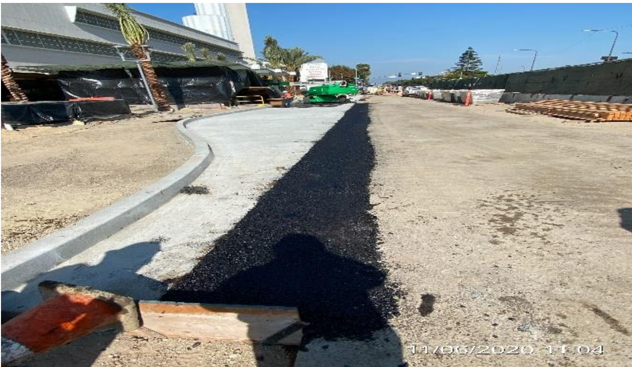
MLK STATION – Placing asphalt concrete around the bus pad pay on the east side of the plaza.
