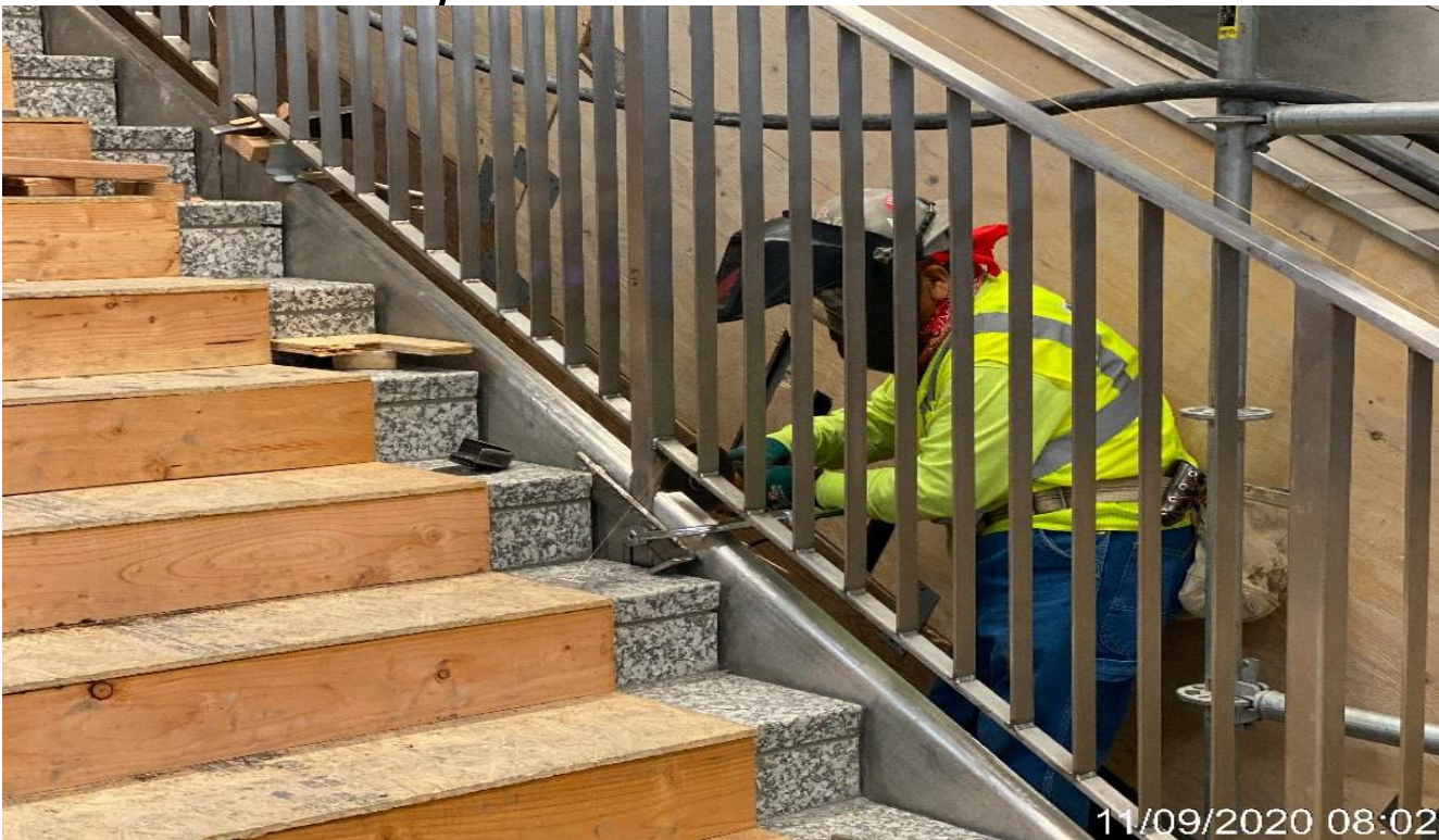
LEIMERT PARK STATION – Continue installing/welding guardrails to Staircases 3&4 from concourse to platform.
