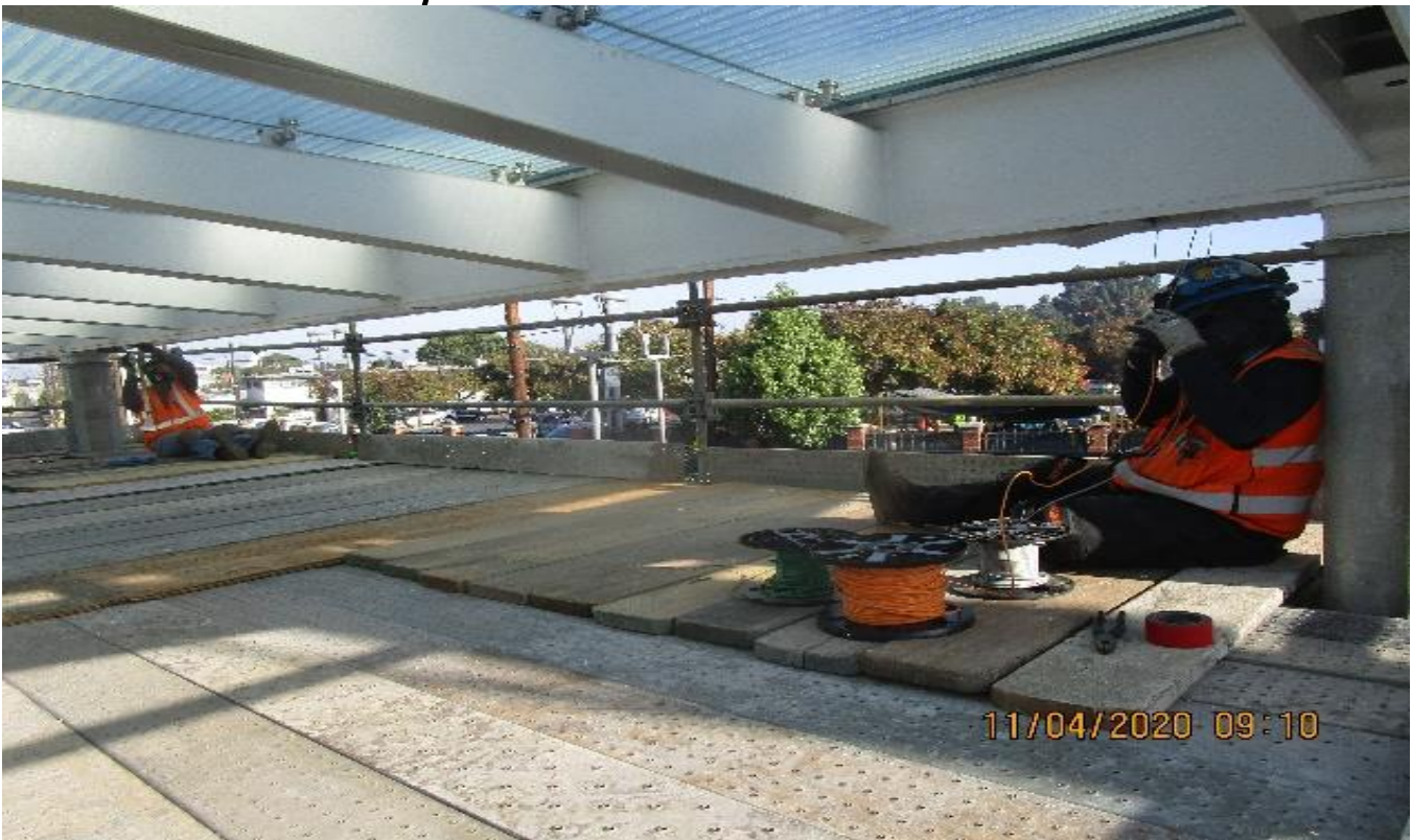
LEIMERT PARK STATION – Drilling holes to the main entrance canopy outriggers for BOCA light fixture installation at the plaza.
