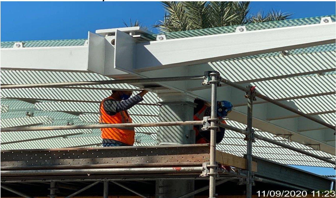
LEIMERT PARK STATION – Continue installing BOCA light fixtures to the main entrance canopy outriggers at the plaza.
