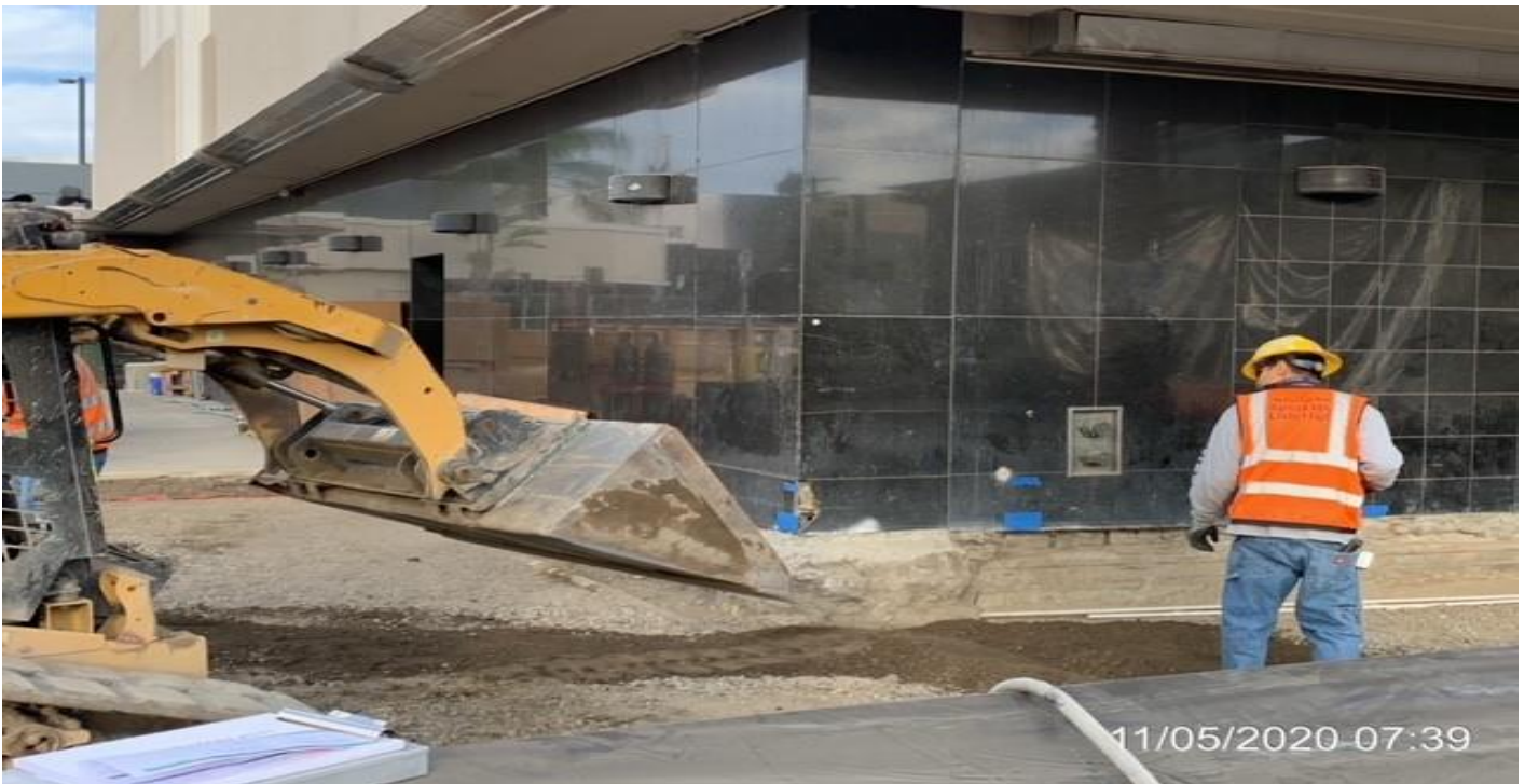
MLK STATION – Backfilling/compacting irrigation trenches at the far northwest area of the plaza.
