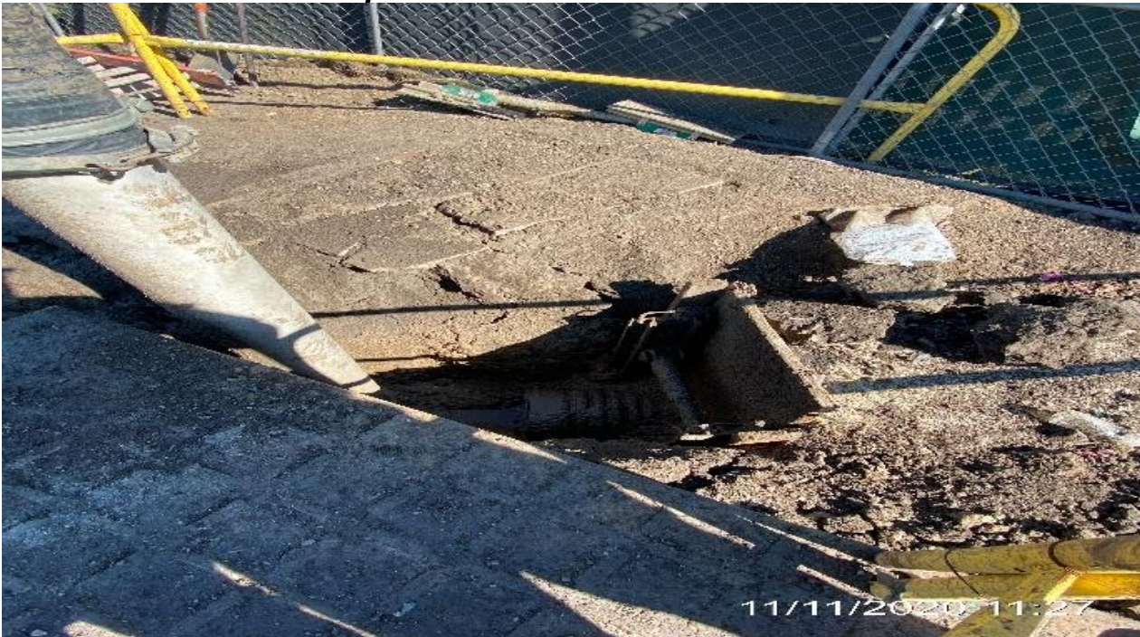
PARK MESA – Continue excavating and installing HDPE pipe connection from Catch Basin #6 to TPSS#7 on the northeast corner of Crenshaw Blvd and 60th St.
