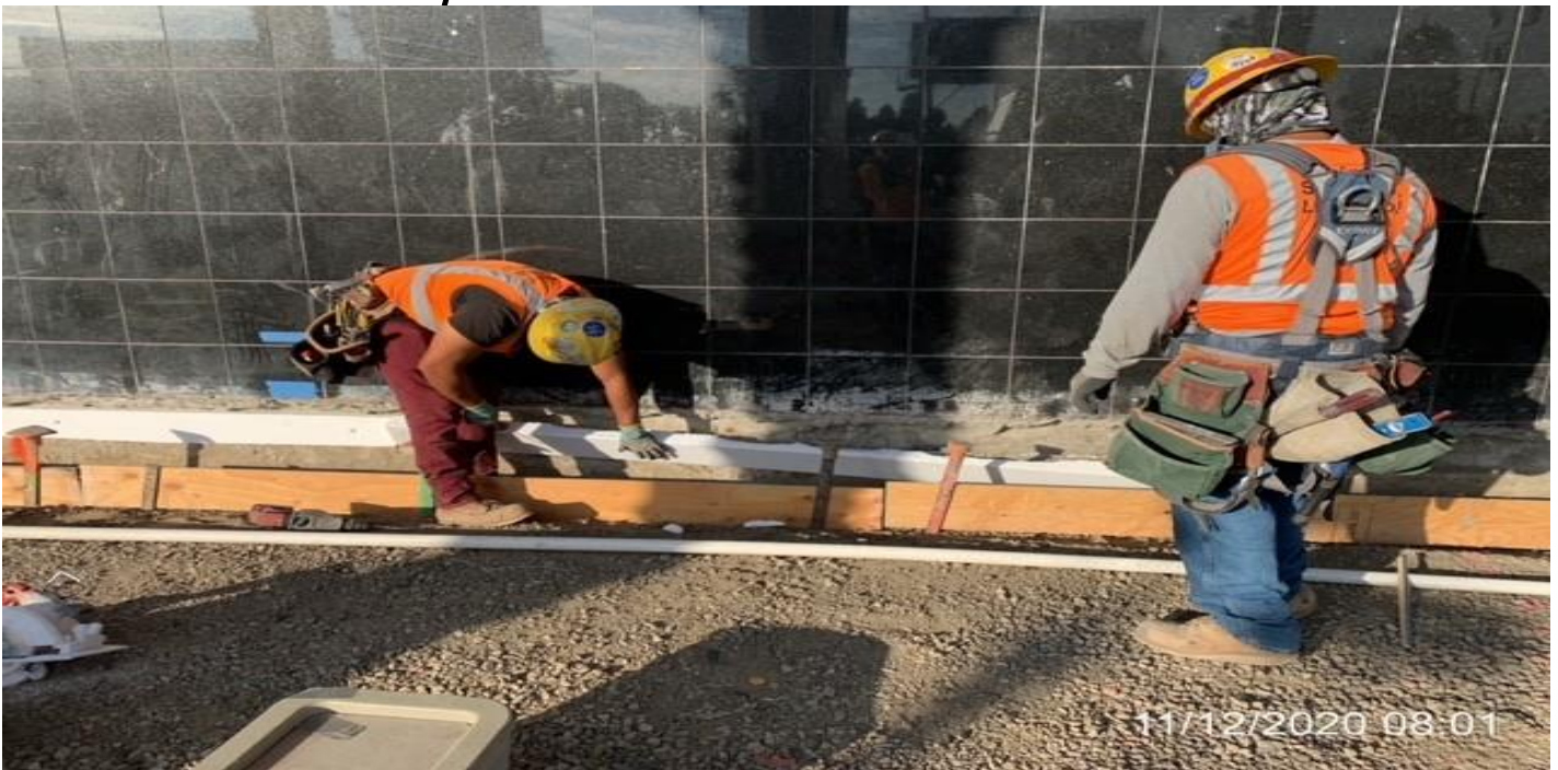
MLK STATION – Setting formwork along the northeast corner of the Mall at the plaza for new walkway curb.
