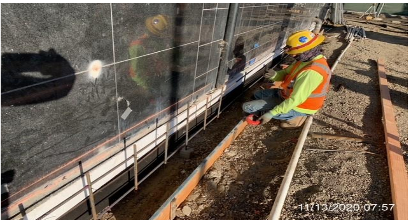
MLK STATION – Continue setting formwork along the northeast corner of the Mall at the plaza for new walkway curb.
