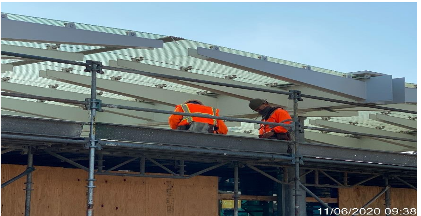
LEIMERT PARK STATION – Installing BOCA light fixtures to the main entrance canopy outriggers at the plaza.
