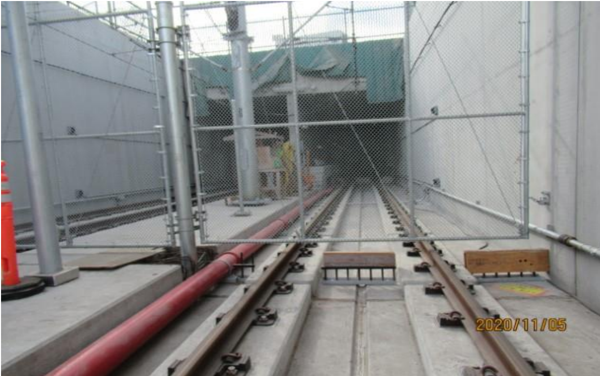
UG3 – UG3 north portal SB track stopping point for field site walk STA 311+48 (looking south).
