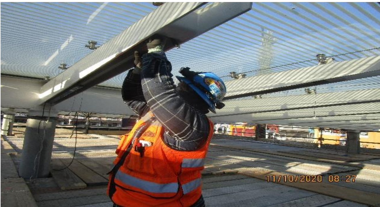
LEIMERT PARK STATION – Continue installing BOCA light fixtures to the main entrance canopy outriggers at the plaza.
