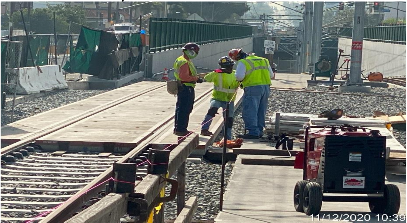
HYDE PARK STATION – Performing layout for guardrail installation for the NB entrance ramp leading to the platform.
