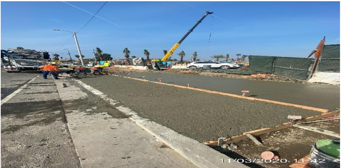
EXPO STATION - Built formwork and placing concrete for sidewalk panels along westbound Obama Blvd and Crenshaw Blvd.
