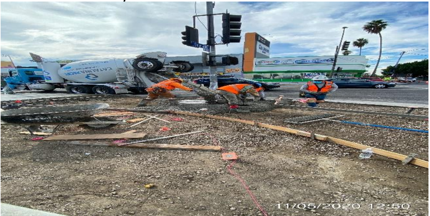
EXPO STATION – Built formwork and placed concrete for new ADA ramp on the southeast corner of Obama Blvd and Crenshaw Blvd.
