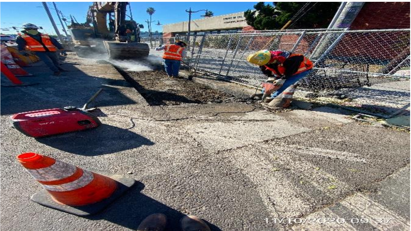
EXPO STATION– Slot paving on southbound Crenshaw Blvd between Obama Blvd and Exposition Blvd.
