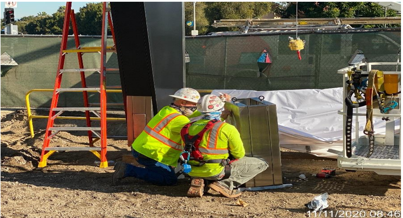
MLK STATION – Installing top cabinet face section to the Grand Pylon Sign at the northeast corner of the plaza.
