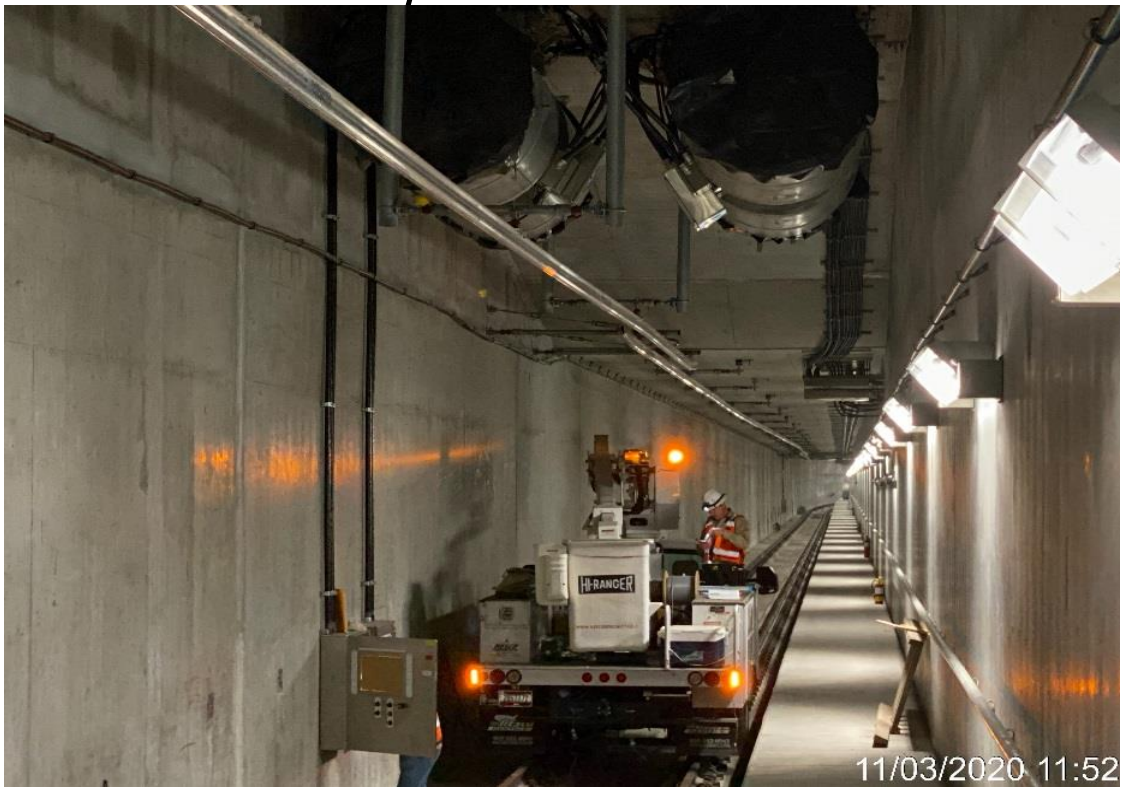
UG3 – Working on tunnel booster fans on the northbound tunnel at STA 292+30.
