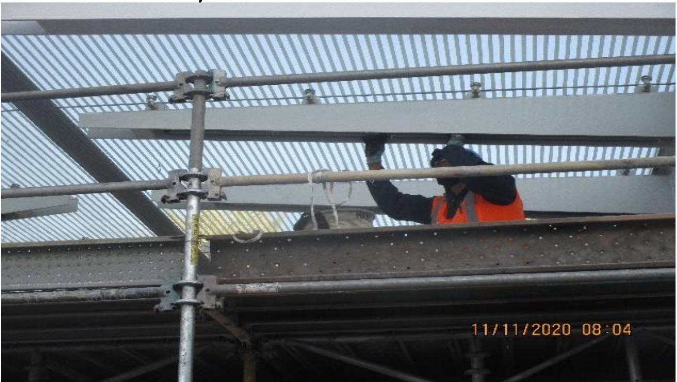
LEIMERT PARK STATION – Continue installing BOCA light fixtures to the main entrance canopy outriggers at the plaza.
