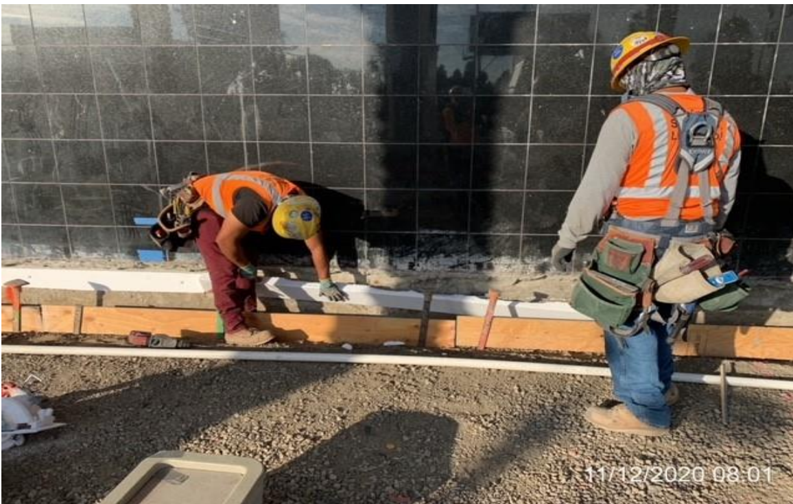
MLK STATION – WSCC crew setting formwork for curb next to mall footing.
