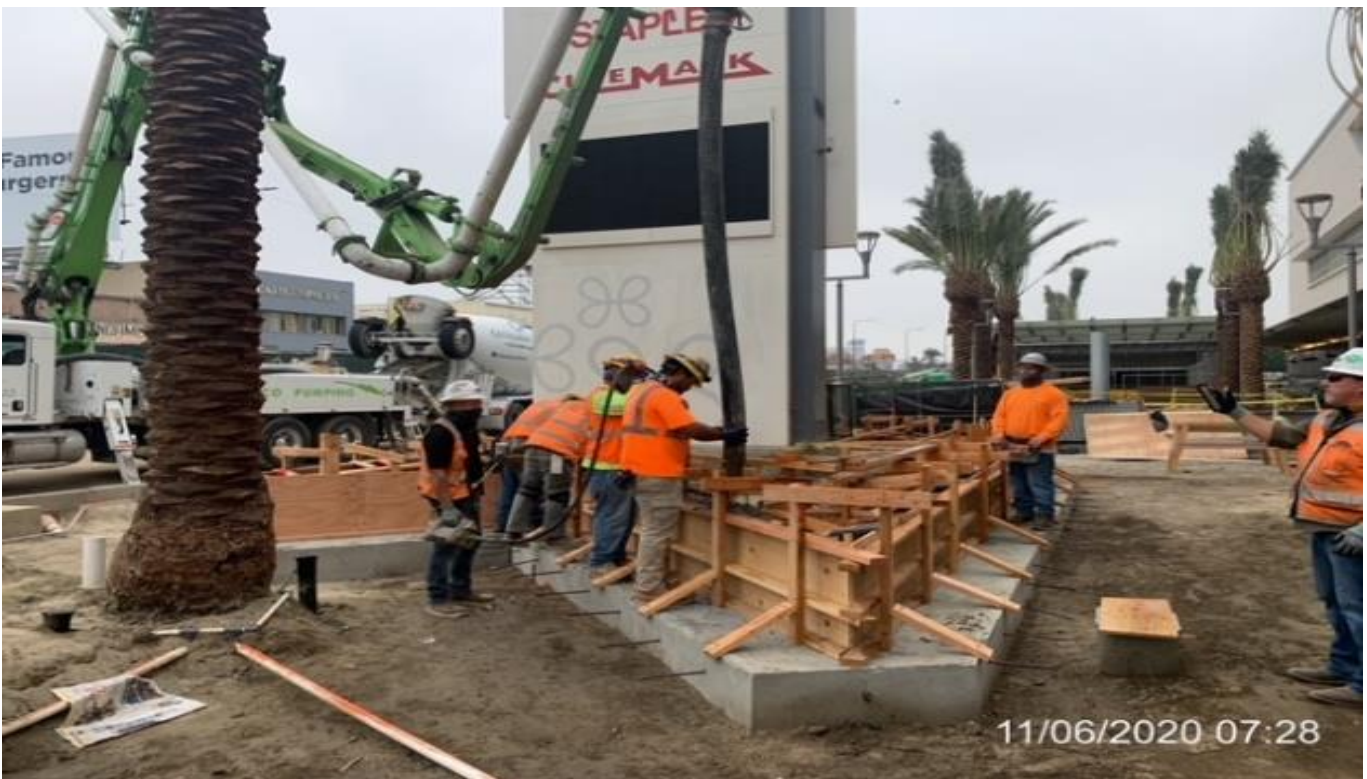
MLK STATION – Placing concrete for the north planter wall at the plaza.
