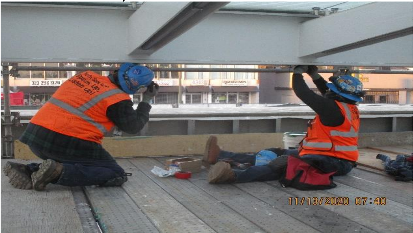
LEIMERT PARK STATION – Continue installing BOCA light fixtures to the main entrance canopy outriggers at the plaza.
