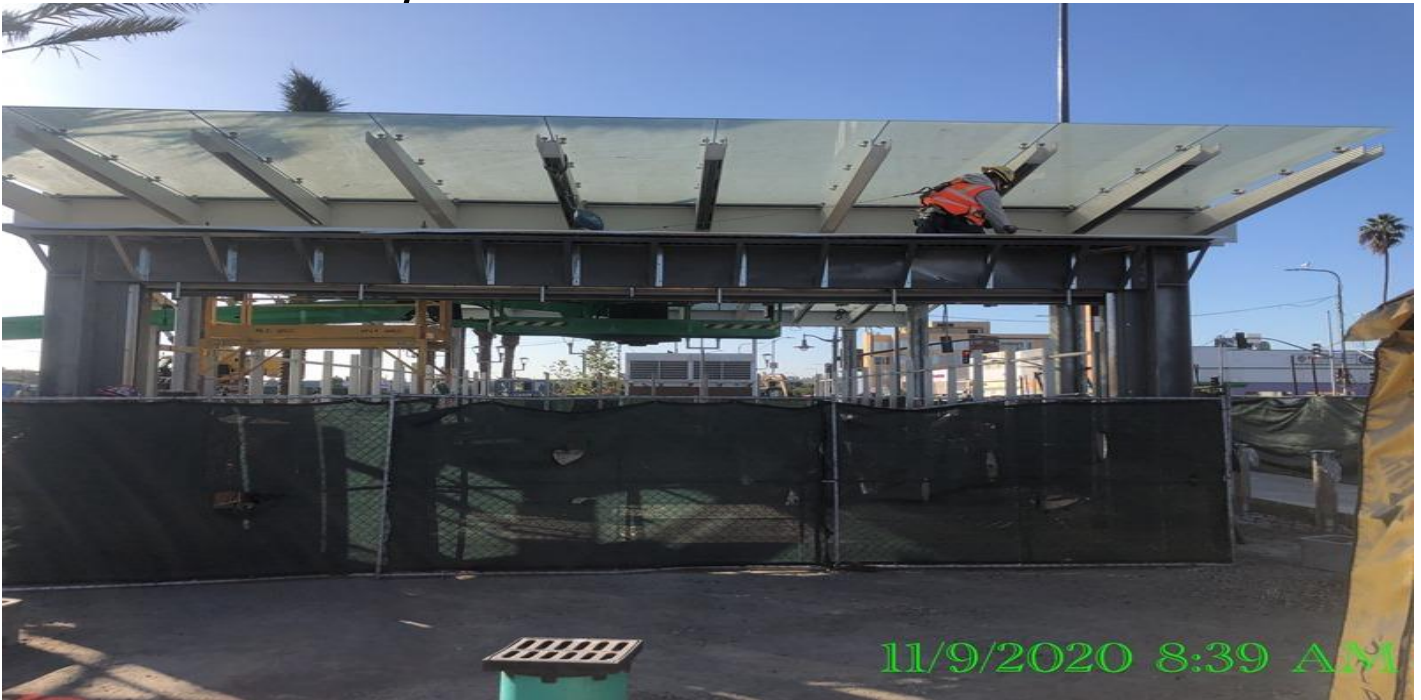
EXPO STATION – Continue installing BOCA light fixtures to the main entrance canopy outriggers at the plaza.
