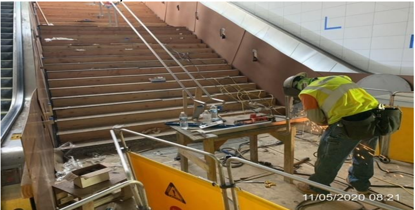
MLK STATION – Continue installing center handrail for Staircase 1 from plaza to concourse.
