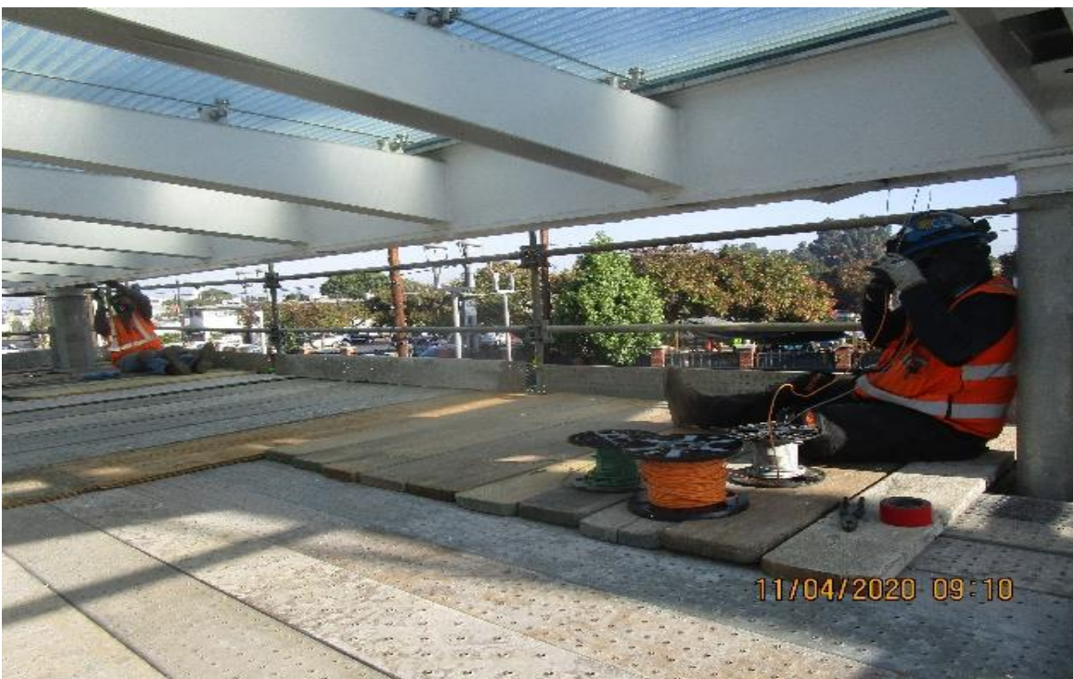
Leimert Park – Vernon Plaza, Entrance Canopy begin pulling #10 XHHW-2 for normal & emergency lighting fixtures.
