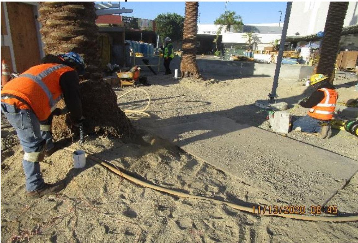
MLK STATION – MLK (S) Plaza, begin pulling #12 XHHW-2 landscape lighting wiring at palm trees to embedded pull boxes
