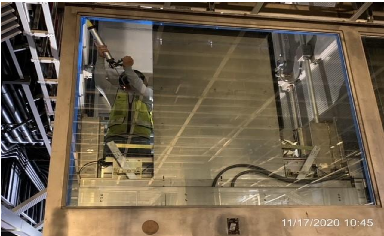
EXPO STATION – Caulking and sealing glass panels for Elevators 3&4 at the platform.
