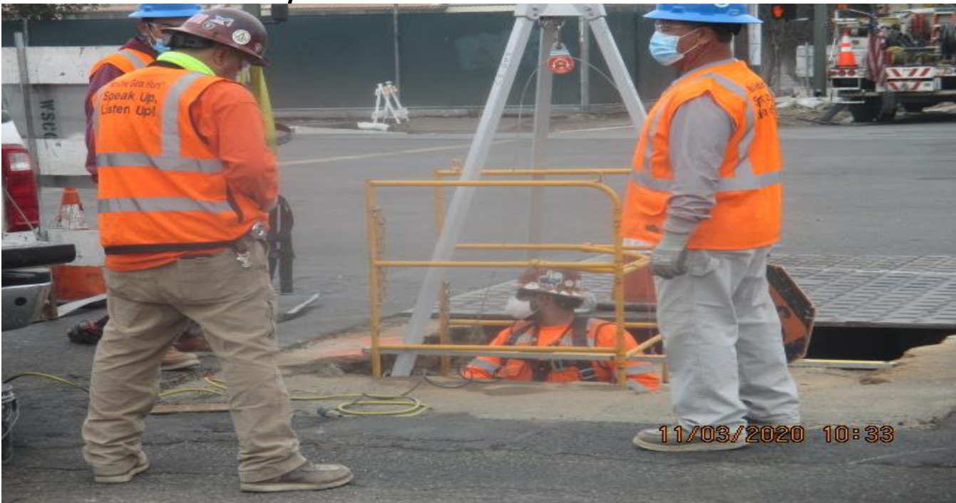
PARK MESA – Continue sacking and patching and installing ladder rungs to Manhole #20 on northbound Crenshaw Blvd and 60th St.
