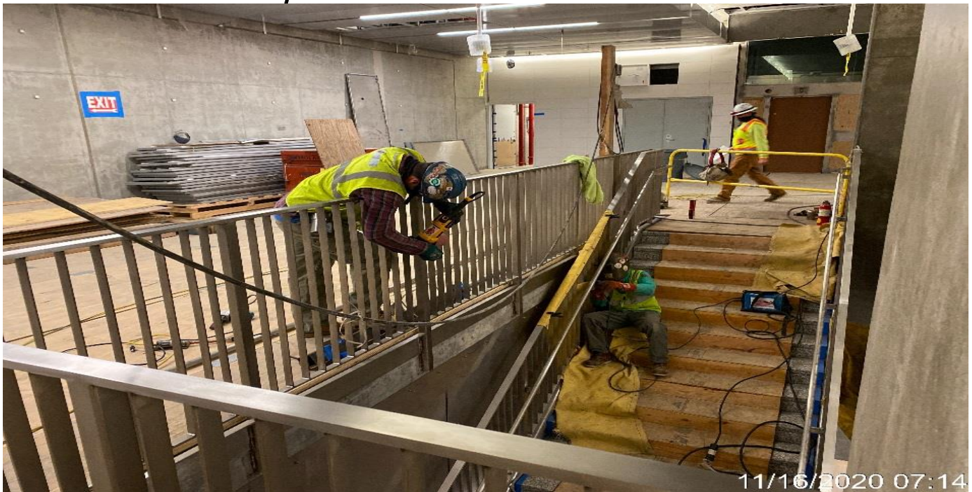
LEIMERT PARK STATION – Continue installing/welding guardrails to Staircases 3 from concourse to platform.
