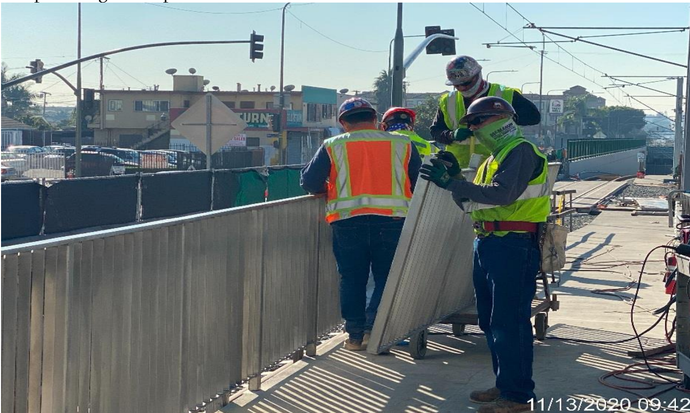
HYDE PARK STATION – Installing guardrails along the NB entrance ramp leading into the platform.
