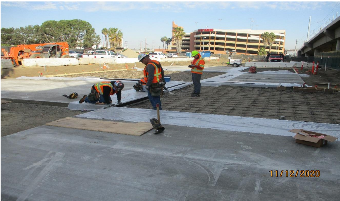
AVIATION/CENTURY- Setting expansion board for the plaza hardscape at the Aviation Station.
