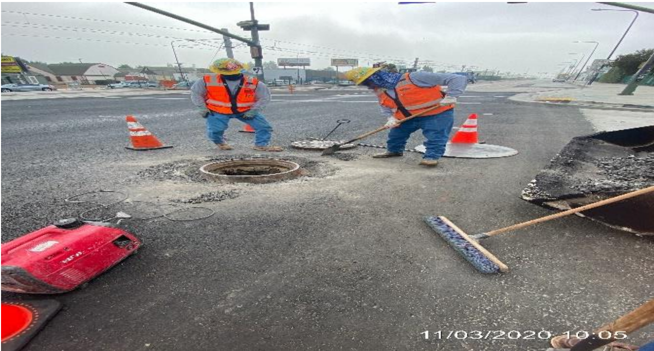
PARK MESA – Removing rings and access covers of sewer maintenance holes in preparation for final grind and overlay of north and southbound Crenshaw Blvd and 48th St.
