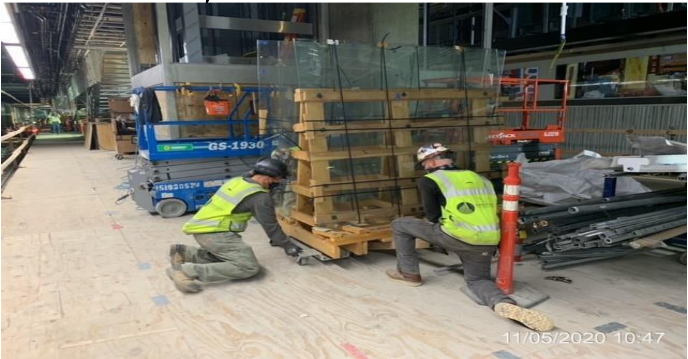
EXPO STATION – Mobilizing glass panels to install to Elevators 3&4 at the platform.
