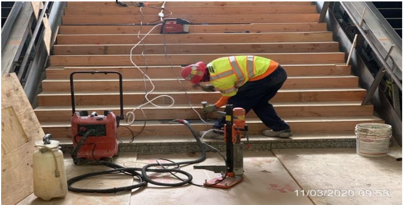
EXPO STATION – Coring for center handrail installation at Staircase 1 from plaza to concourse.
