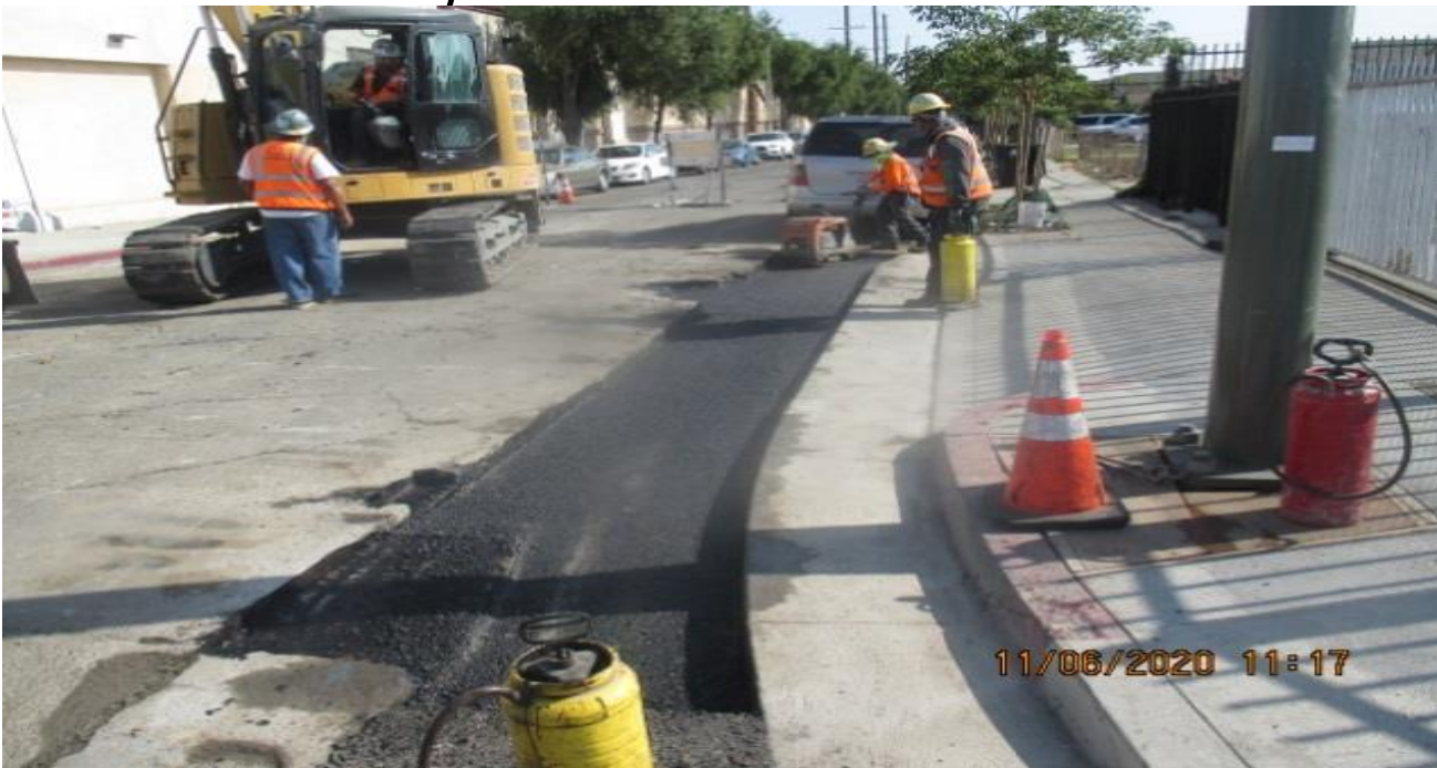
PARK MESA – Placed asphalt concrete on the southeast corner of Crenshaw Blvd and 59th St.
