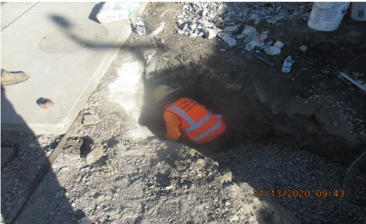
PARK MESA – Excavating and installing for HDPE pipe connection from Catch Basin #6 to TPSS#7 on the northeast corner of Crenshaw Blvd and 60th St.
