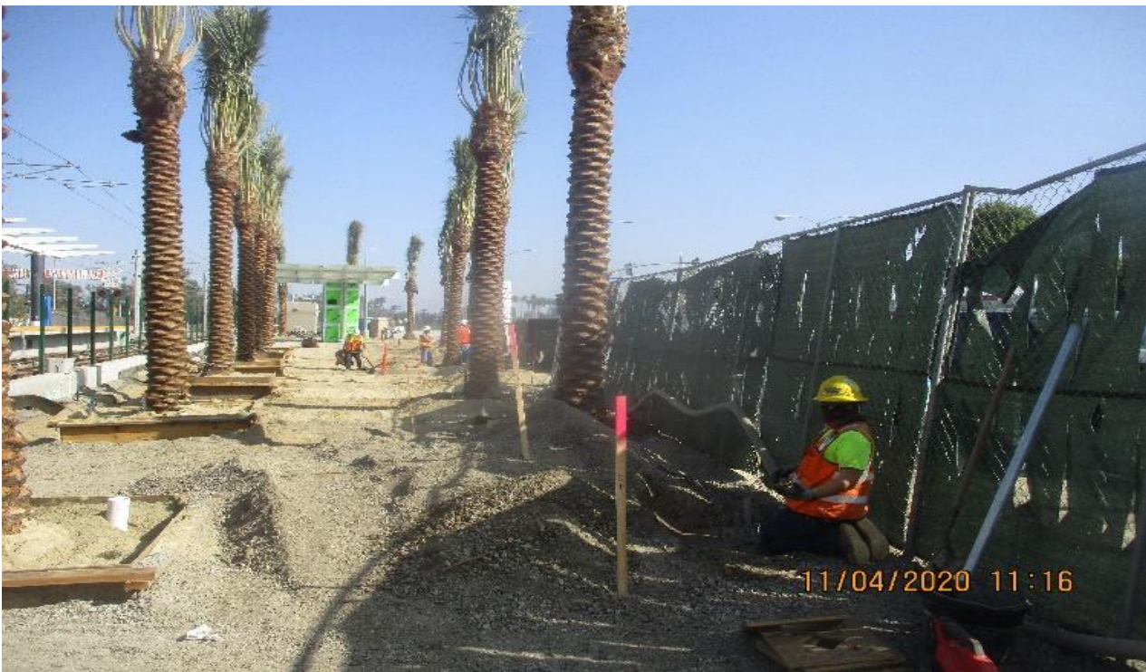
La Brea – WSCC Prepare To place light poles on foundations at La Brea Plaza
