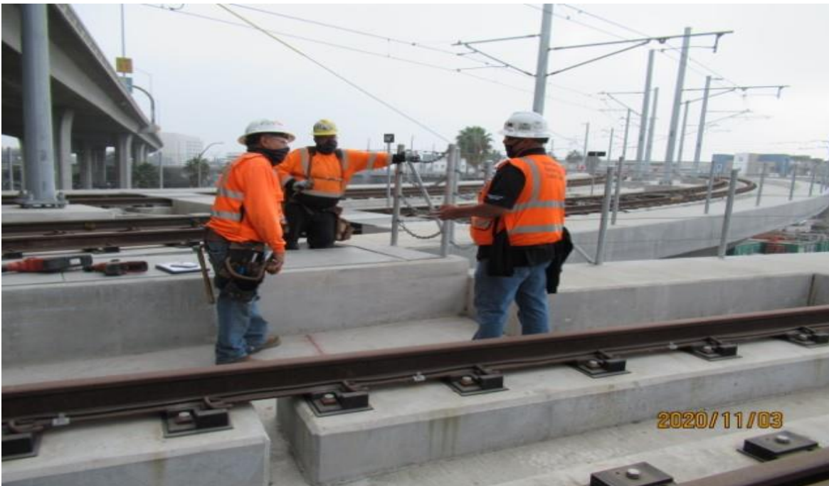
Guideway- WSCC working on extending Emergency Walkway crossing at intersection of east & west legs of Wye STA 13+14 (looking east) Rework
