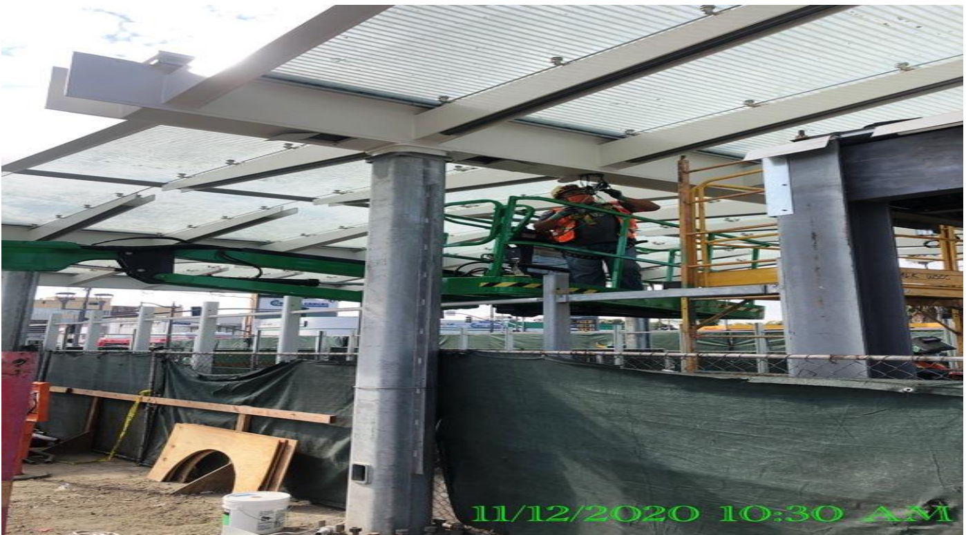
EXPO STATION – Continue installing BOCA light fixtures to the main entrance canopy outriggers at the plaza.
