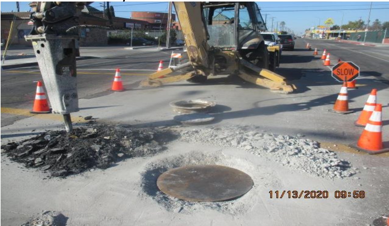
PARK MESA – Removing rings and access covers of sewer maintenance holes and placing protective plates prior to grind and overlay on southbound Crenshaw Blvd and Slauson Ave.
