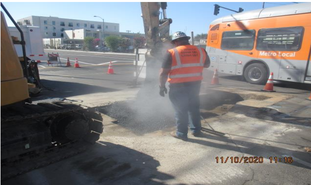
PARK MESA – Placing asphalt concrete around Manhole #20 on northbound Crenshaw Blvd and 60th St.
