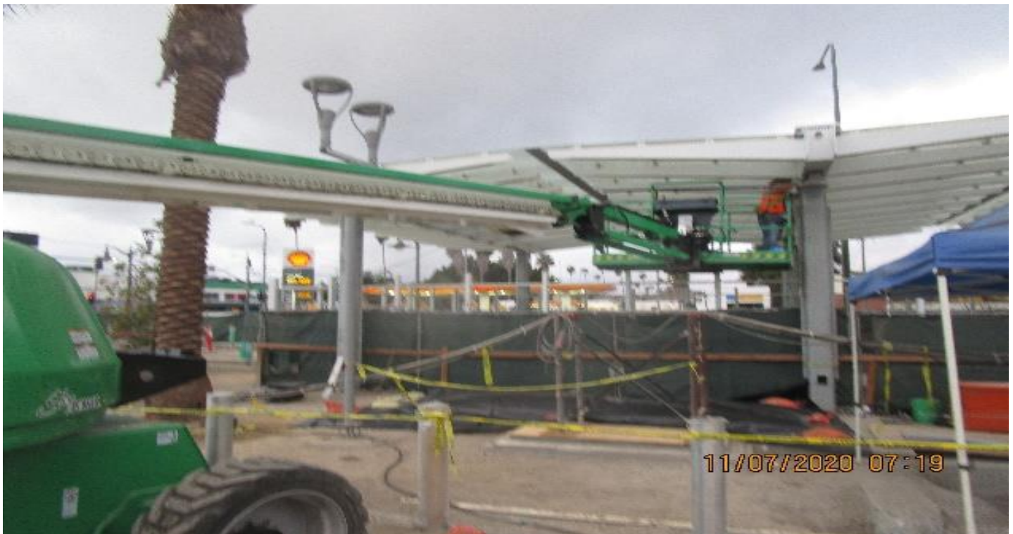
EXPO STATION – Installing BOCA light fixtures to the main entrance canopy outriggers at the plaza.
