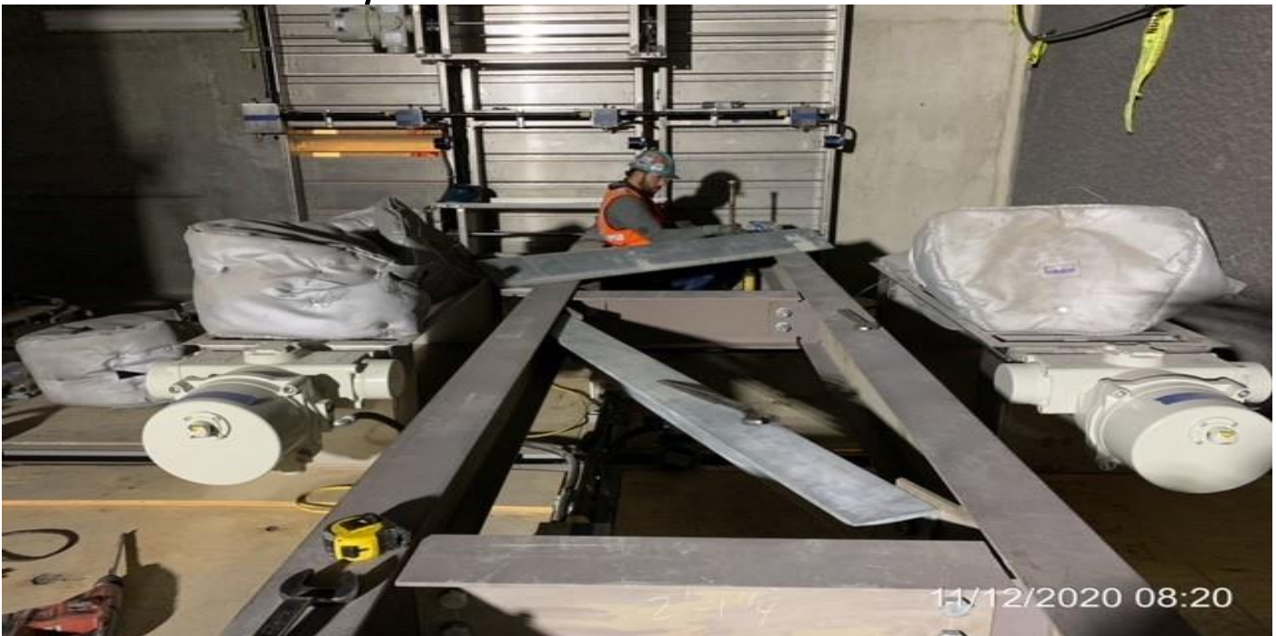
MLK STATION – Installing metal framing for catwalk installation in the Tunnel Vent/OTE Plenum North C-143 at the concourse.
