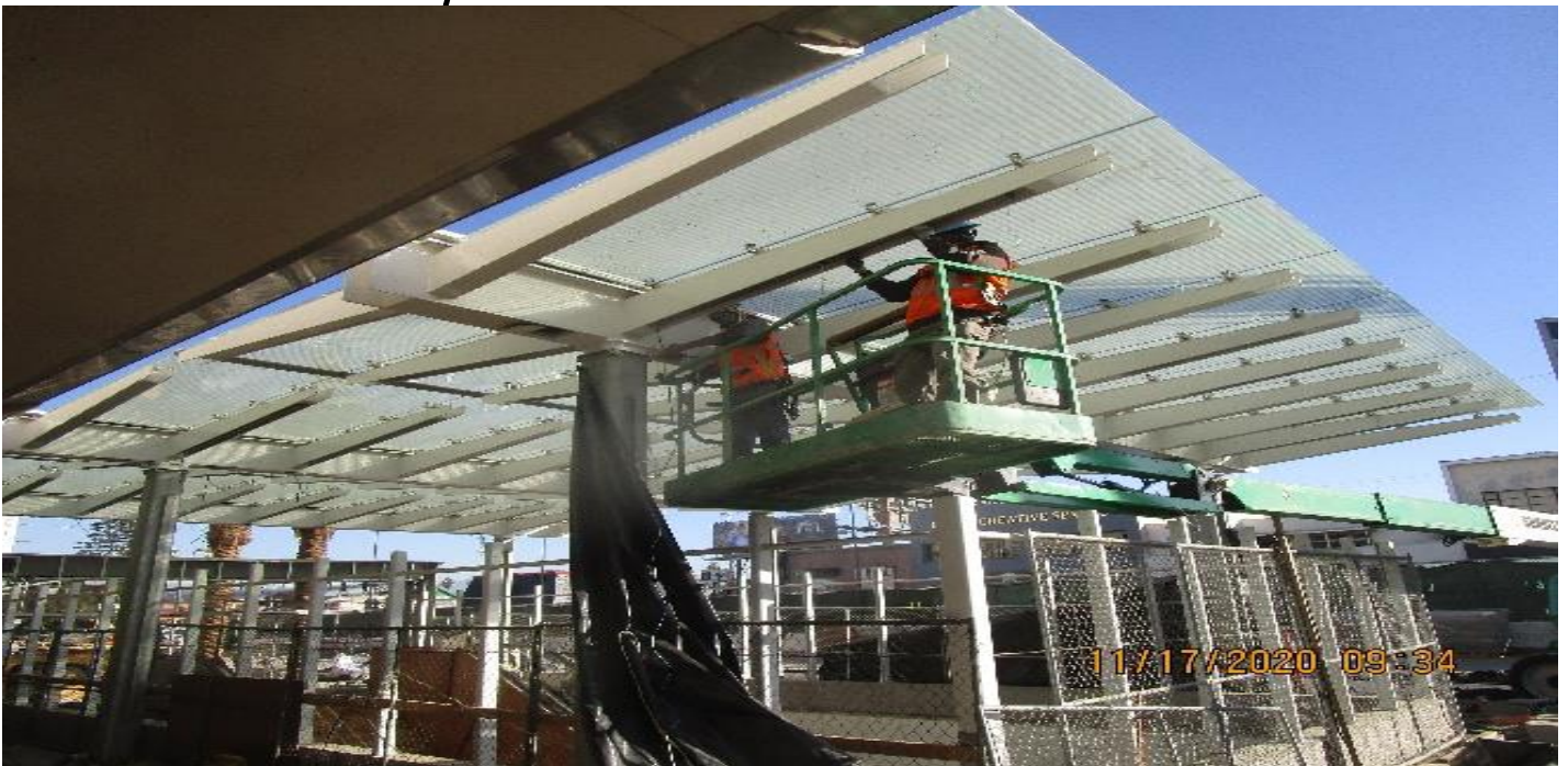
MLK STATION – Installing BOCA light fixtures to the main entrance canopy outriggers at the plaza.
