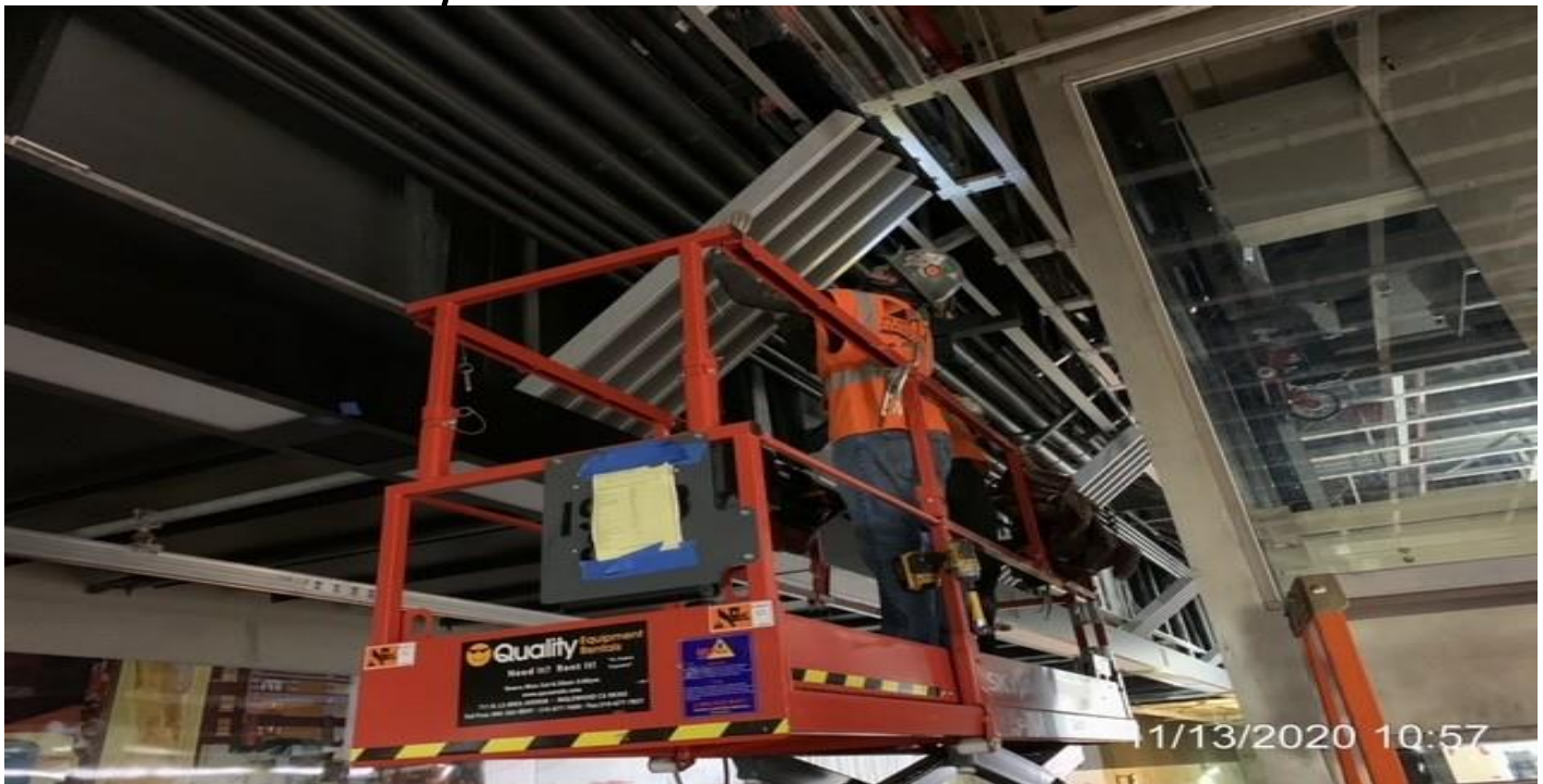
EXPO STATION – Continue installing diagonal screen panels along the northbound and southbound side of the platform.
