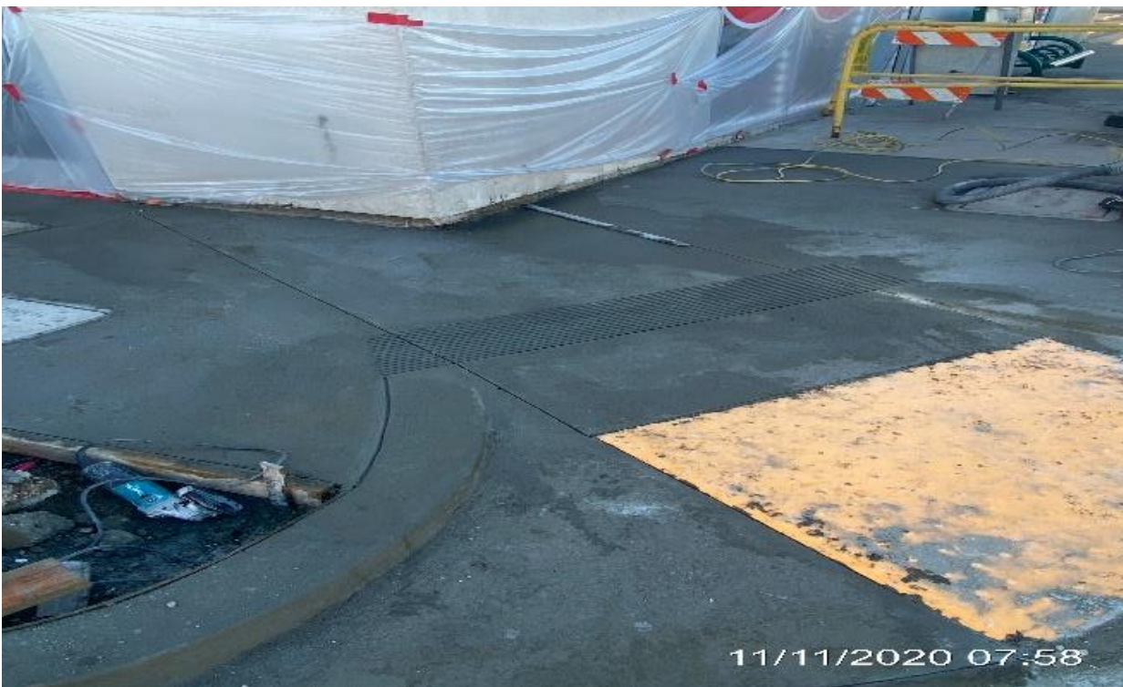
UG3 – Saw cutting ADA ramp and sidewalk installation on the southeast corner of Hyde Park Blvd and Crenshaw Blvd.
