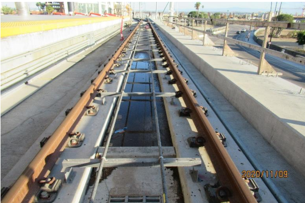
AVIATION/CENTURY- Century/Aviation bridge station platform NB track approx. STA 68+45 ponding storm water inside bridge deck invert (looking north)
