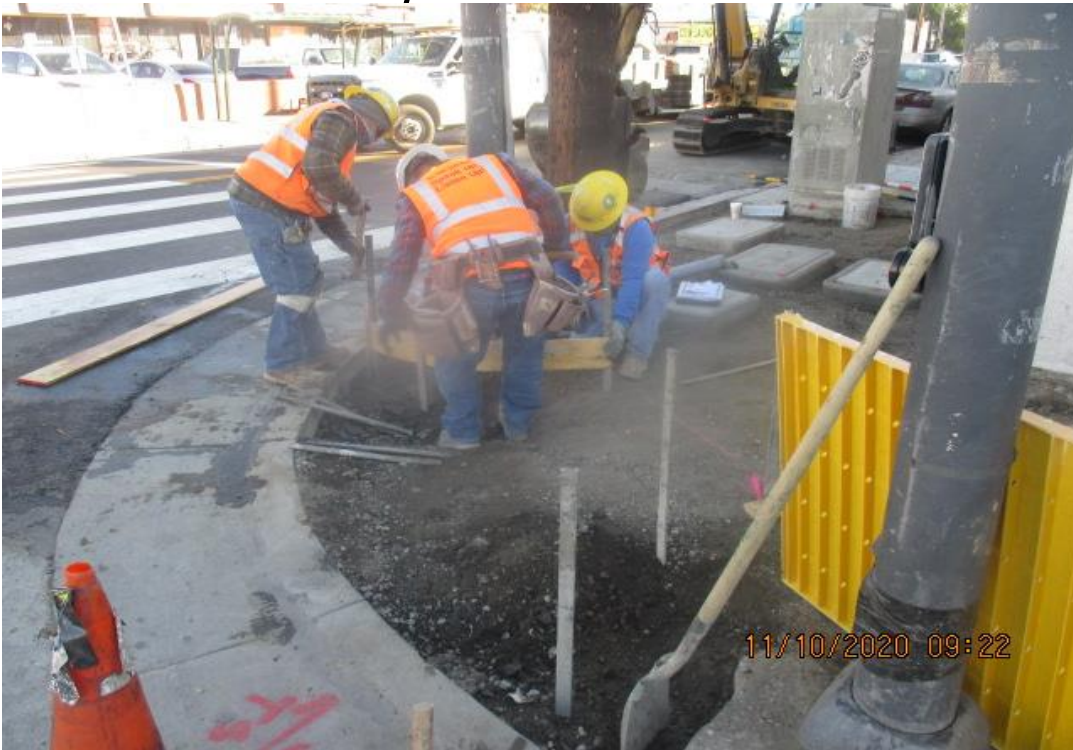
UG3 – Building formwork for new ADA ramp and sidewalk installation on the southeast corner of Hyde Park Blvd and Crenshaw Blvd.
