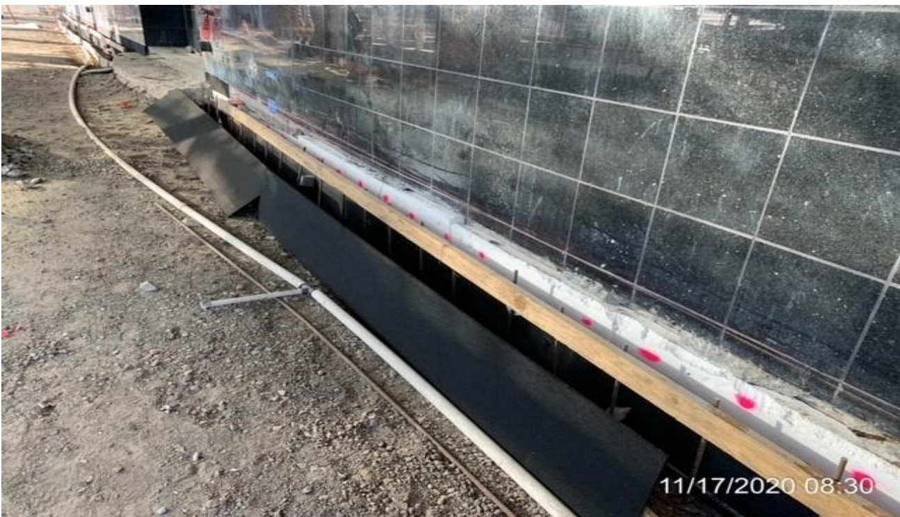
MLK STATION – Installing expansion board for curb wall along the east side of the Mall at the plaza.
