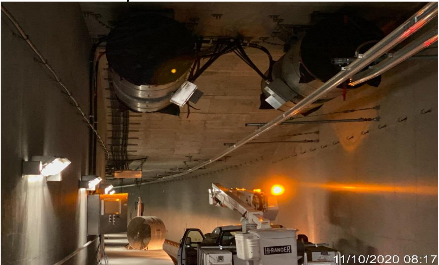
LEIMERT PARK STATION – Working on tunnel booster fans on the northbound tunnel at STA 374+00.
