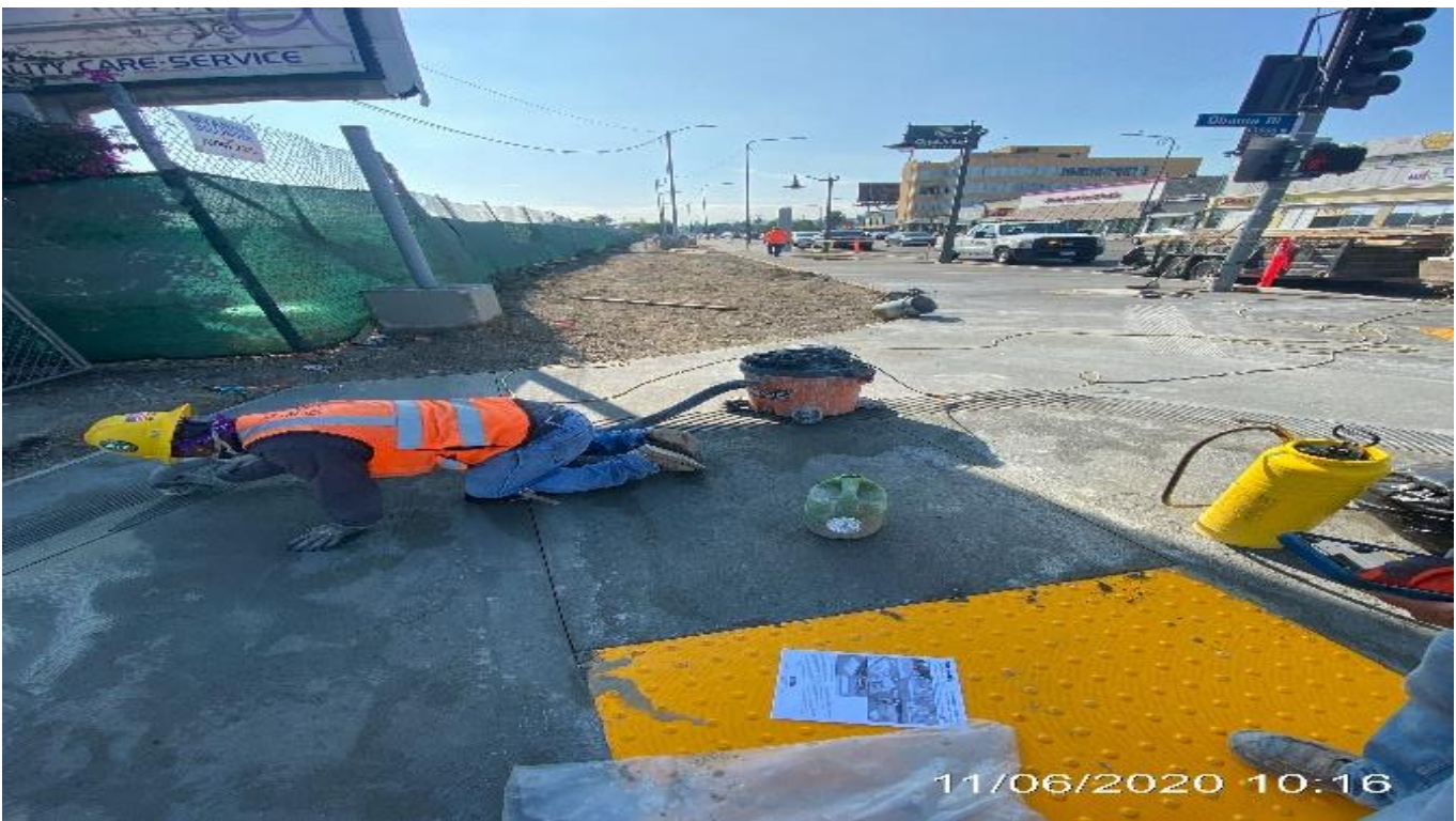
EXPO STATION – Saw cut sidewalk panels and ADA ramp along northbound Crenshaw Blvd and at the southeast corner of Obama Blvd.
