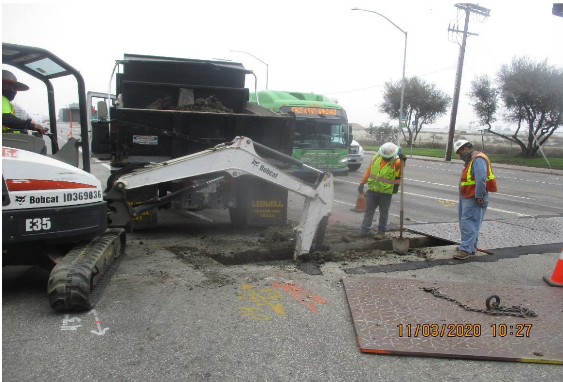
AVIATION/CENTURY- DB Electric Excavate trench for conduit across Aviation at Imp Hwy
