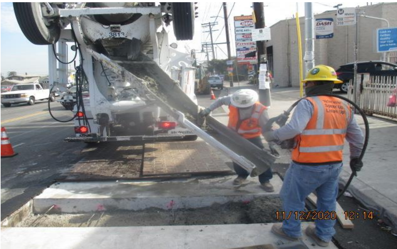
PARK MESA – Placed rebar and concrete for bus pad section on the southeast corner of Crenshaw Blvd and Slauson Ave.
