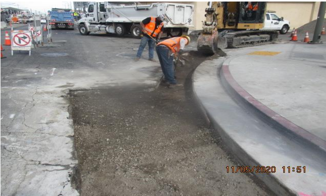
PARK MESA – Saw-cut and excavate along curb radius for asphalt concrete placement on the southeast corner of Crenshaw Blvd and 59th St.
