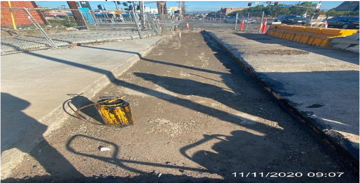
EXPO STATION – Preparing to slot paved remaining section on southbound Crenshaw Blvd between Obama Blvd and Exposition Blvd.
