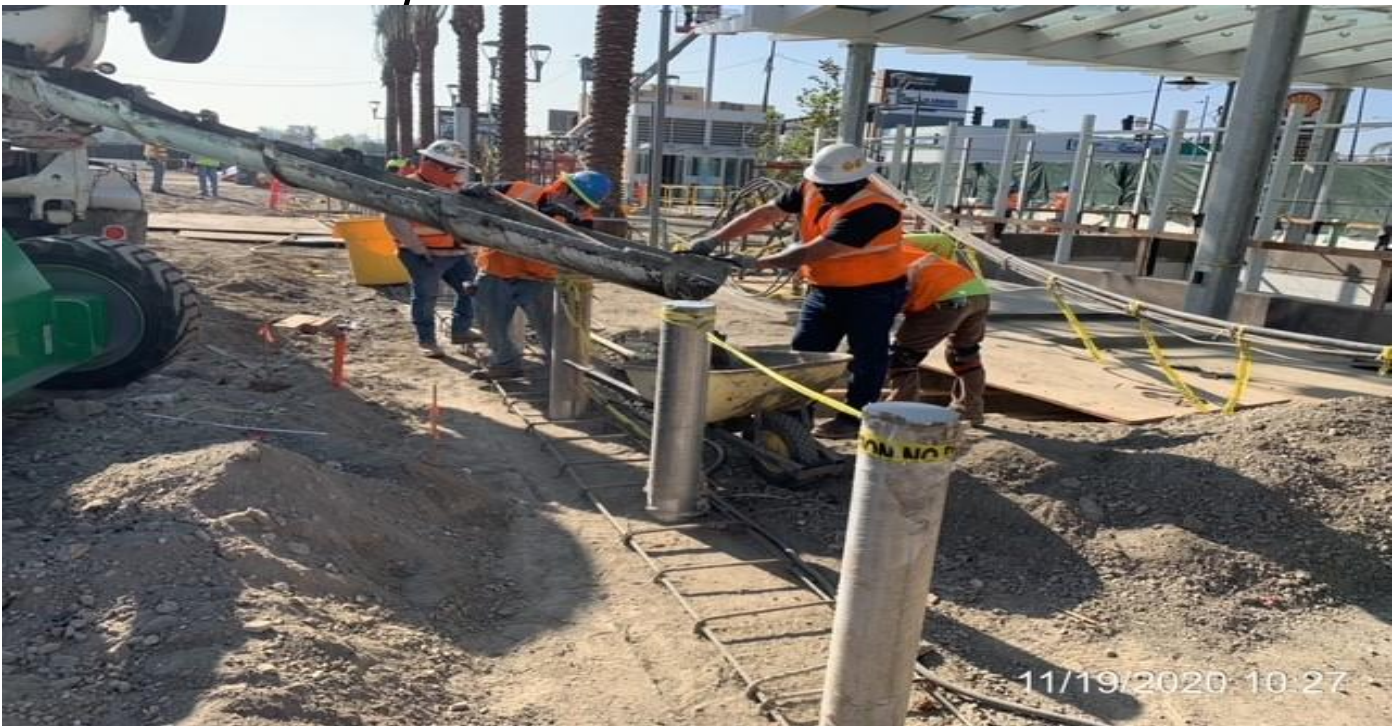
EXPO STATION – Placing concrete over conduit adjacent to the east side bollards at the plaza.
