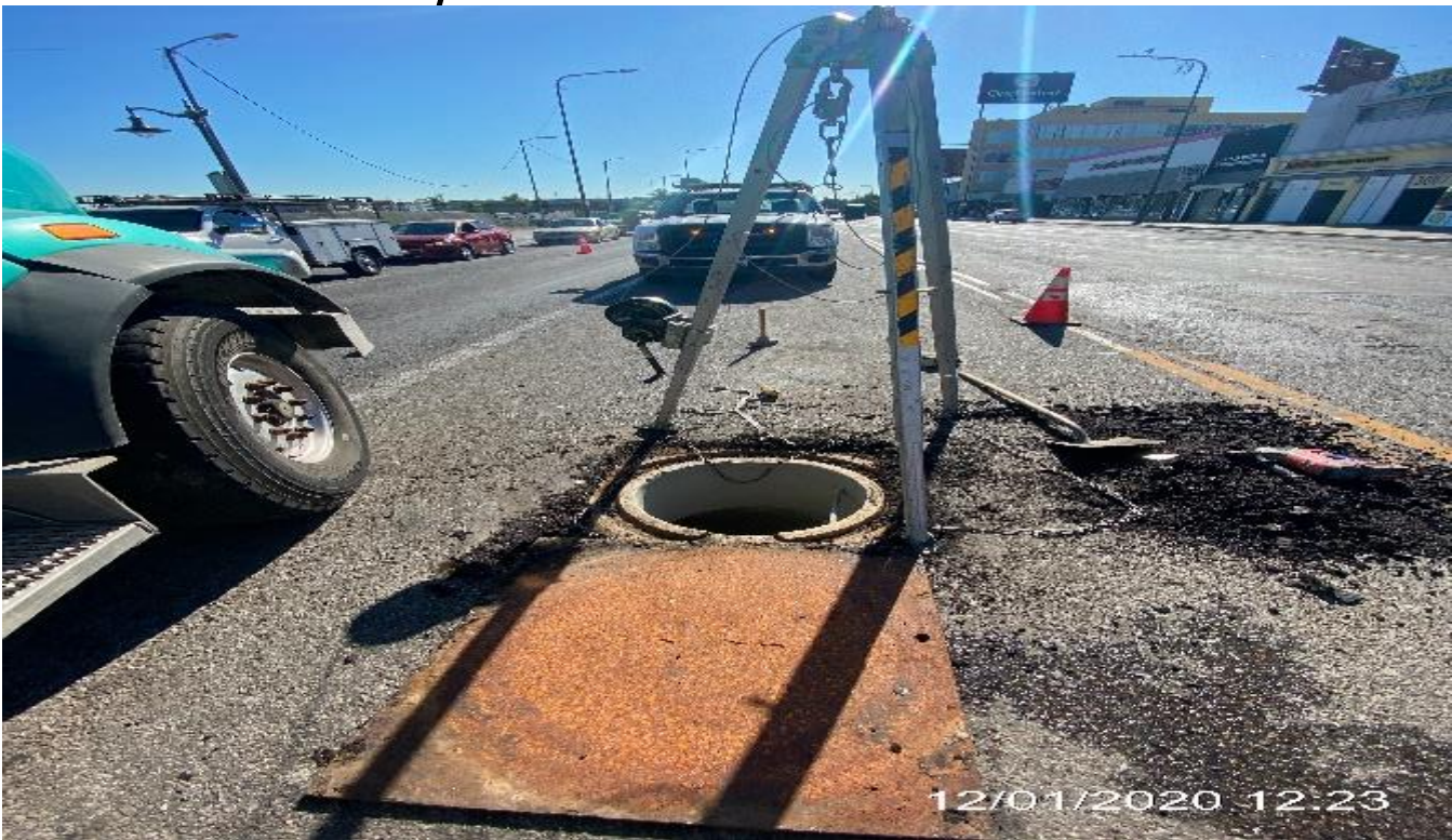
EXPO STATION – Continue preparing Manhole 1 for final inspection at northbound Crenshaw Blvd and Obama Blvd.
