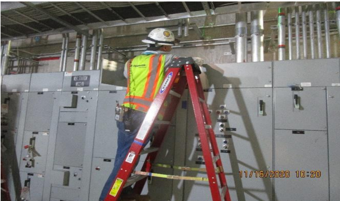
MLK STATION – MLK, Aux power room (N) C132, MCC2/N. resume rough in 18"x18"x12" SCADA PB & (2) 1-1/2" FRC
