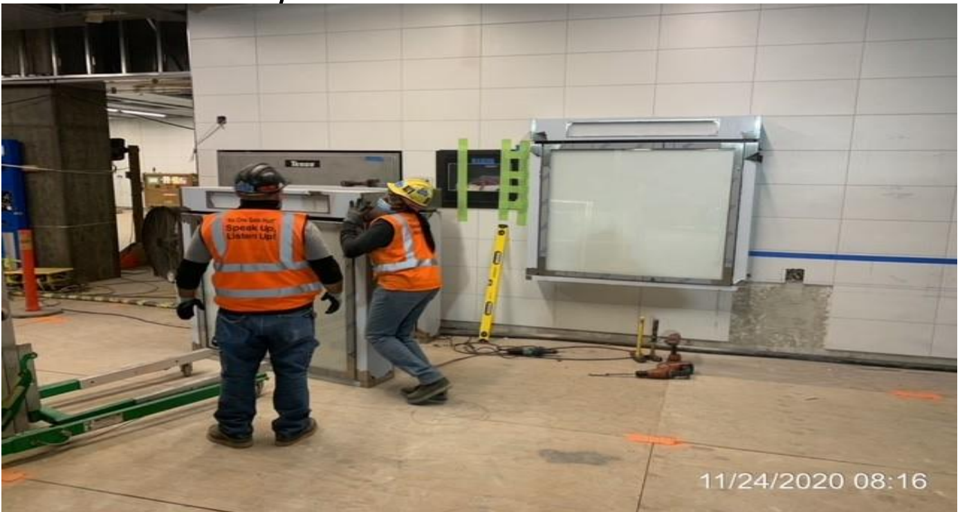
MLK STATION – Installing map cases at the Paid Area of the concourse.
