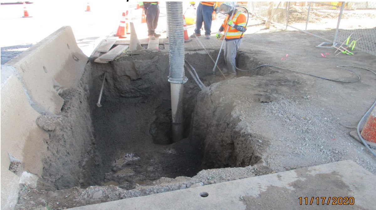
AVIATION/CENTURY- Excavating for the storm drain A catch basing at the SW corner of Aviation and Century.
