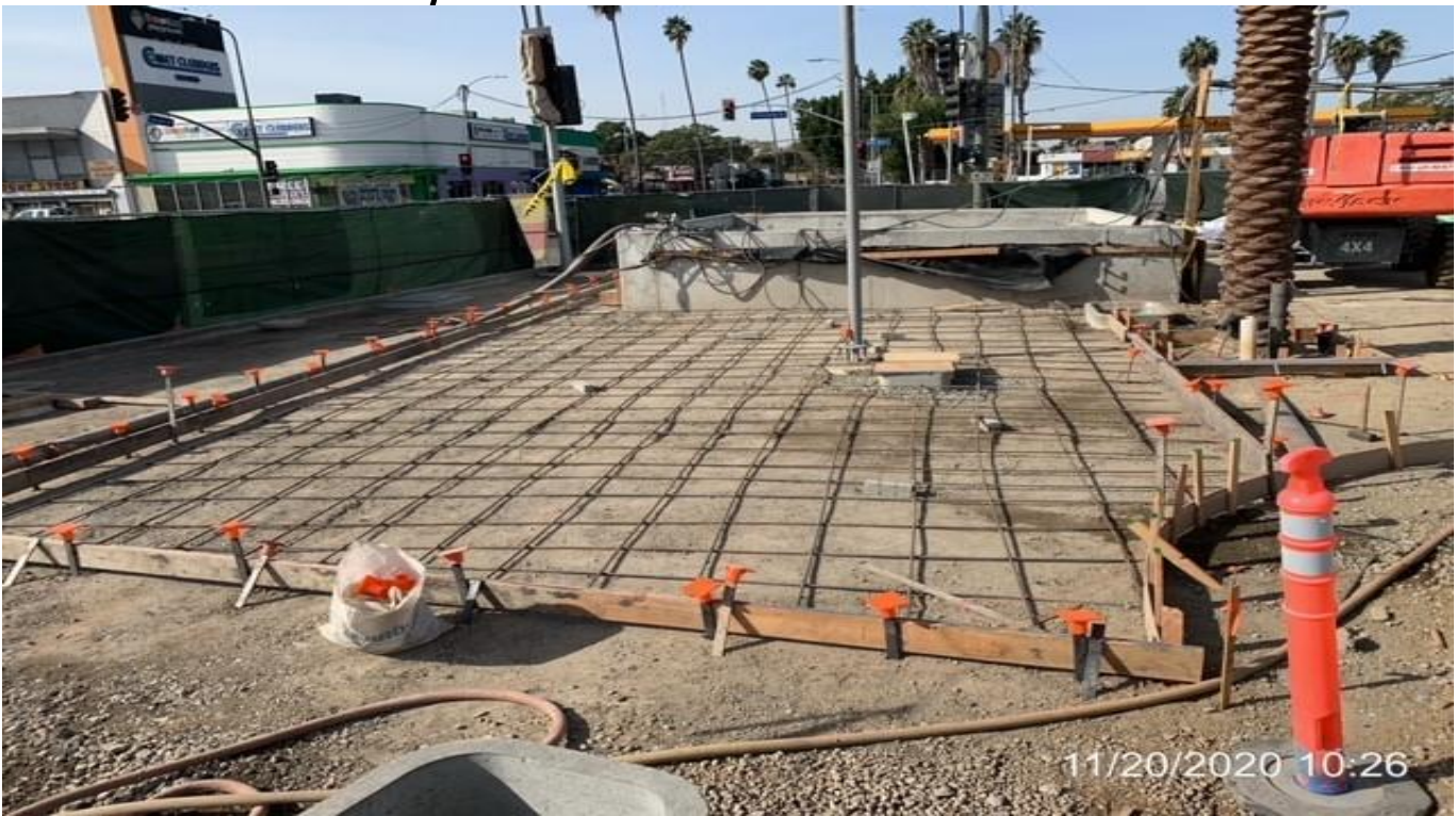
EXPO STATION– Continue building formwork and placing rebar for the architectural topping slab at the south end section of the plaza.
