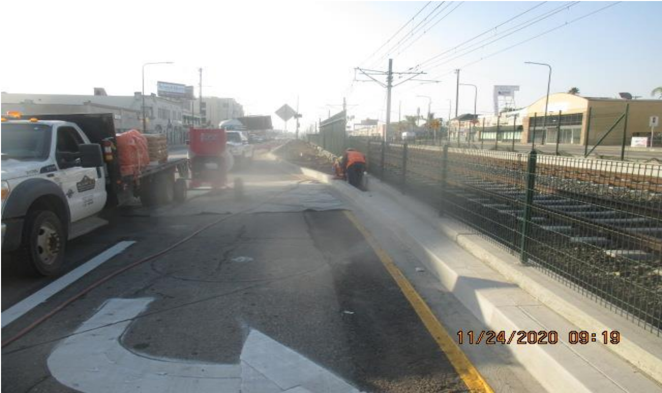
PARK MESA – Continue placing mortar on the northbound median curb on Crenshaw Blvd from 54th St to 52nd St.
