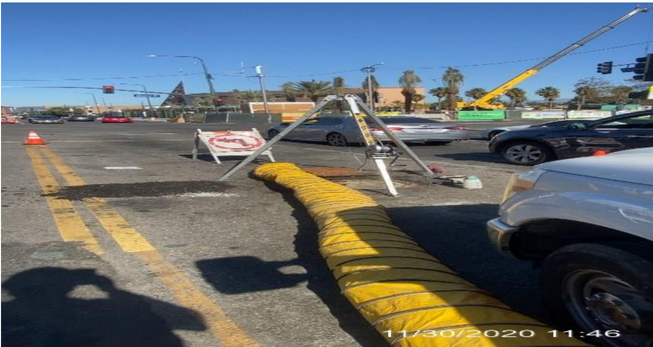
EXPO STATION - Preparing Manhole 1 for final inspection at northbound Crenshaw Blvd and Obama Blvd.
