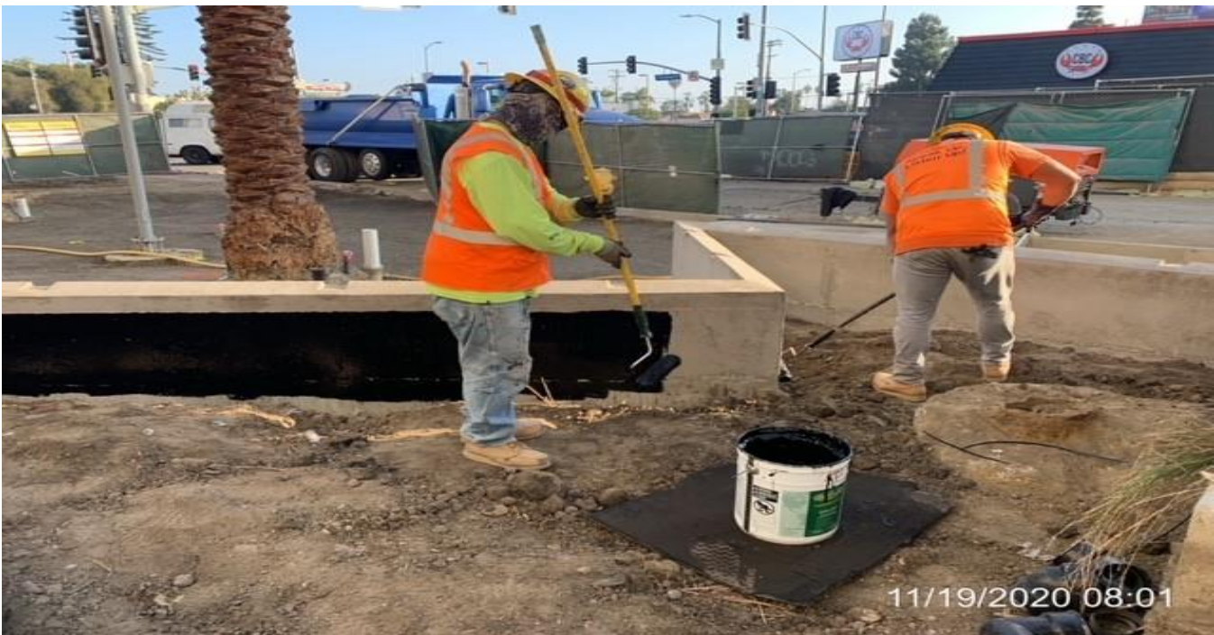
MLK STATION – Applying coat of waterproofing membrane sealant to the interior walls of the north planter at the plaza.
