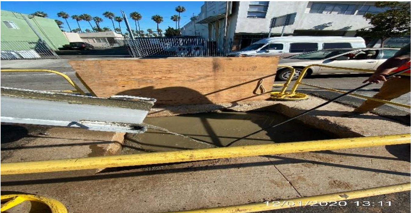
PARK MESA – Placing slurry backfill over pothole on northbound Crenshaw Blvd and 48th St.
