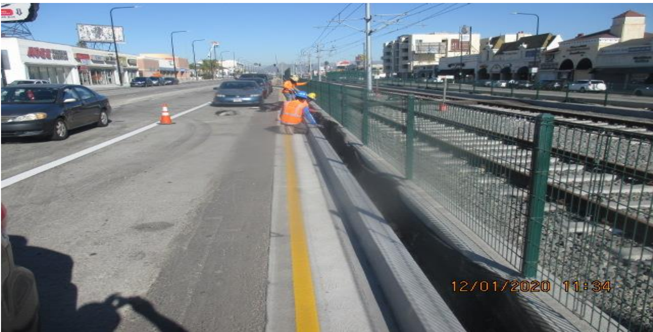
PARK MESA – Continue placing mortar on the southbound median curb on Crenshaw Blvd from 54th St to 52nd St.
