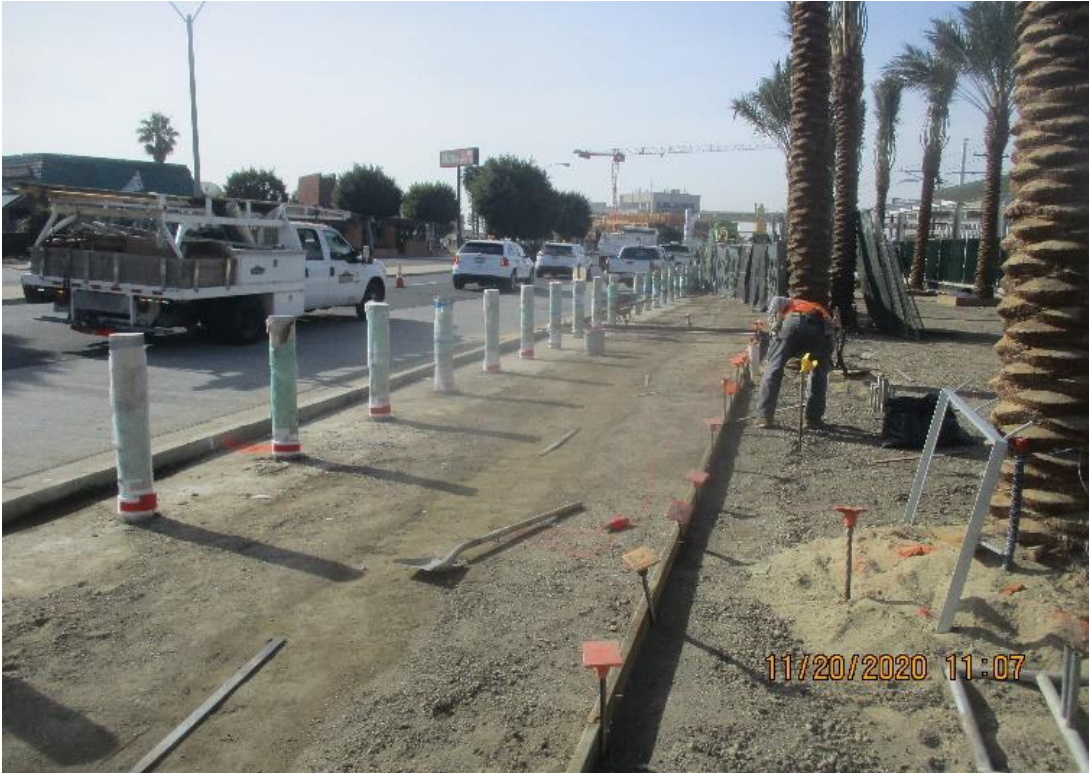
La Brea – WSCC Form and place SWK conc at La Brea Plaza.
