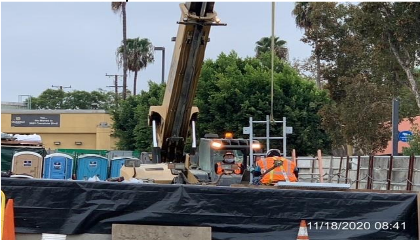
MLK STATION – Lifting steel ladders to be set and installed inside the South Air Exhaust Shaft at the plaza.
