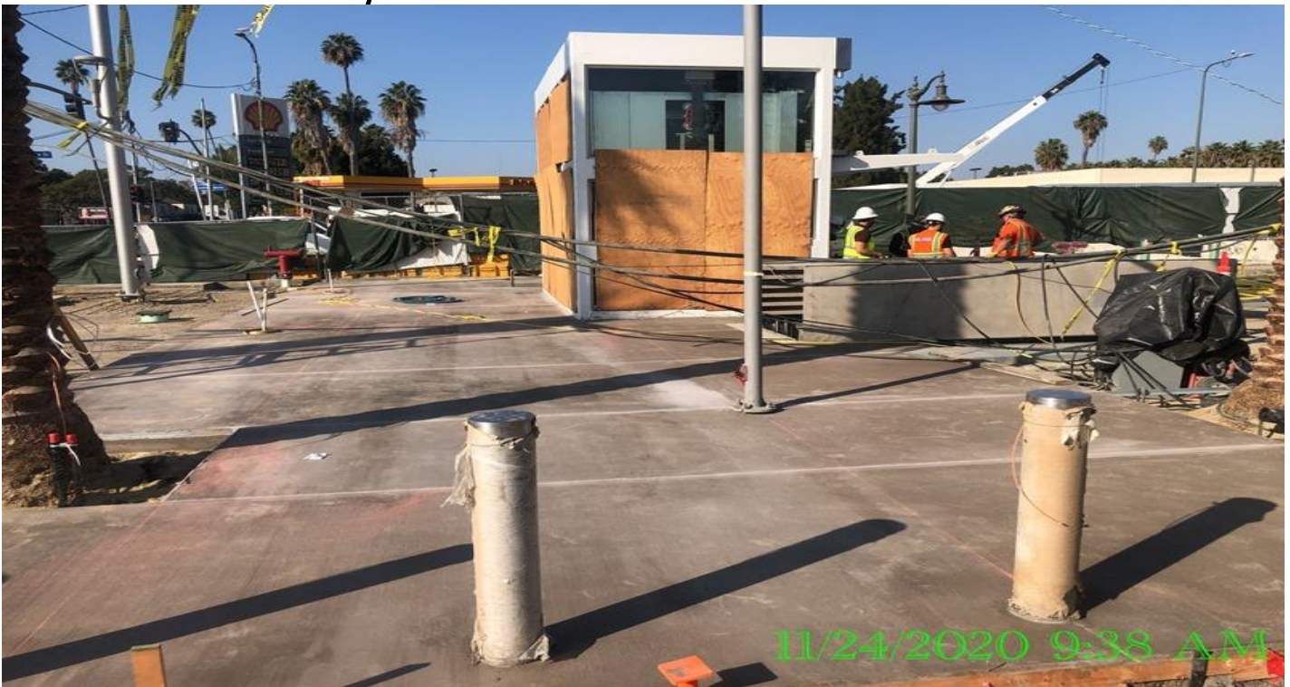
EXPO STATION – Saw cut joints for the architectural topping slab at the south end section of the plaza.
