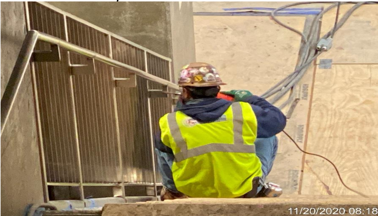
LEIMERT PARK STATION – Continue installing/welding guardrails to Staircases 3 from concourse to platform.
