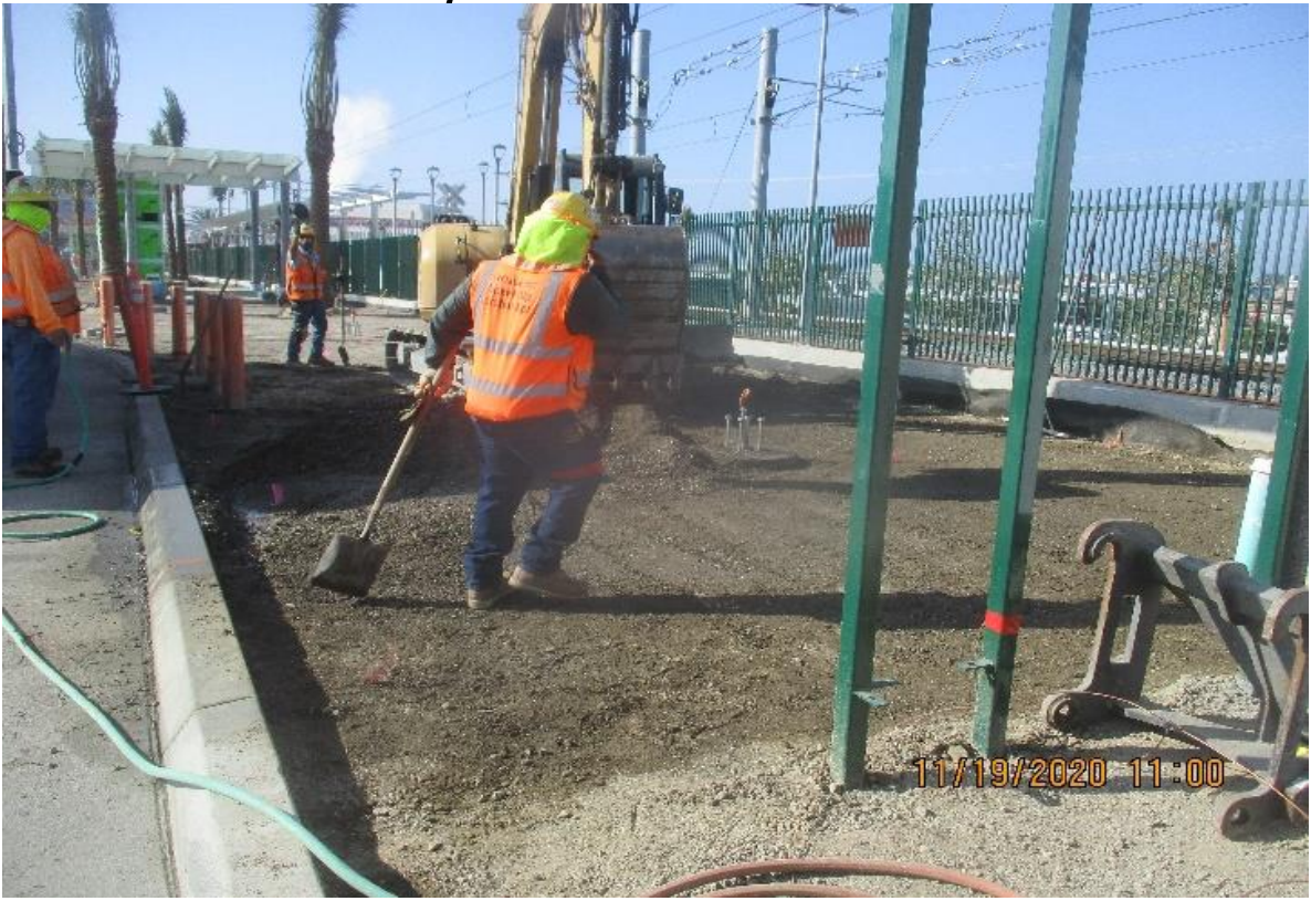
La Brea – WSCC Cut and make grade for SWK at La Brea Plaza.
