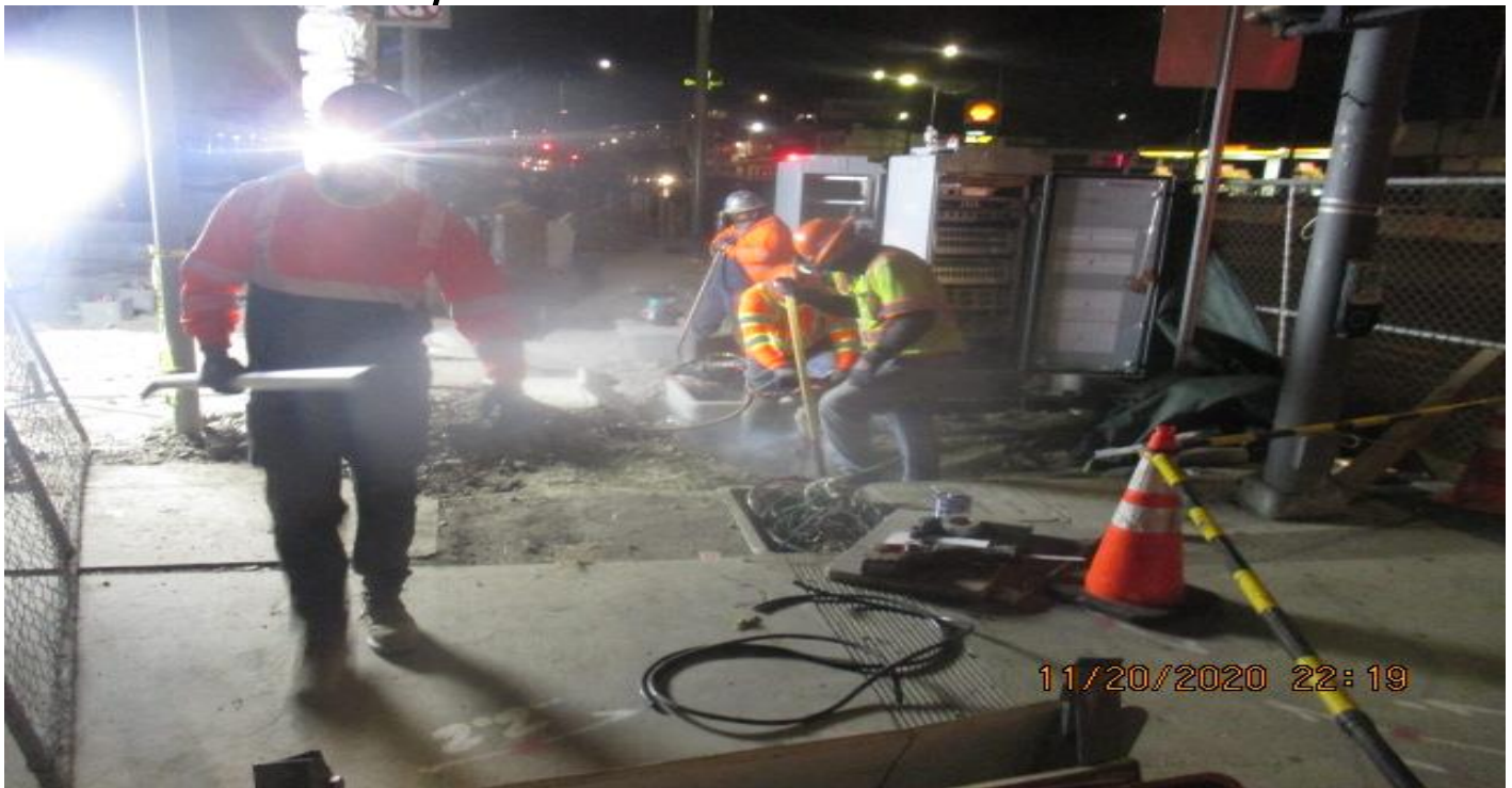
EXPO STATION– Excavating for fiber optic conduit installation at the northwest corner area of the plaza.
