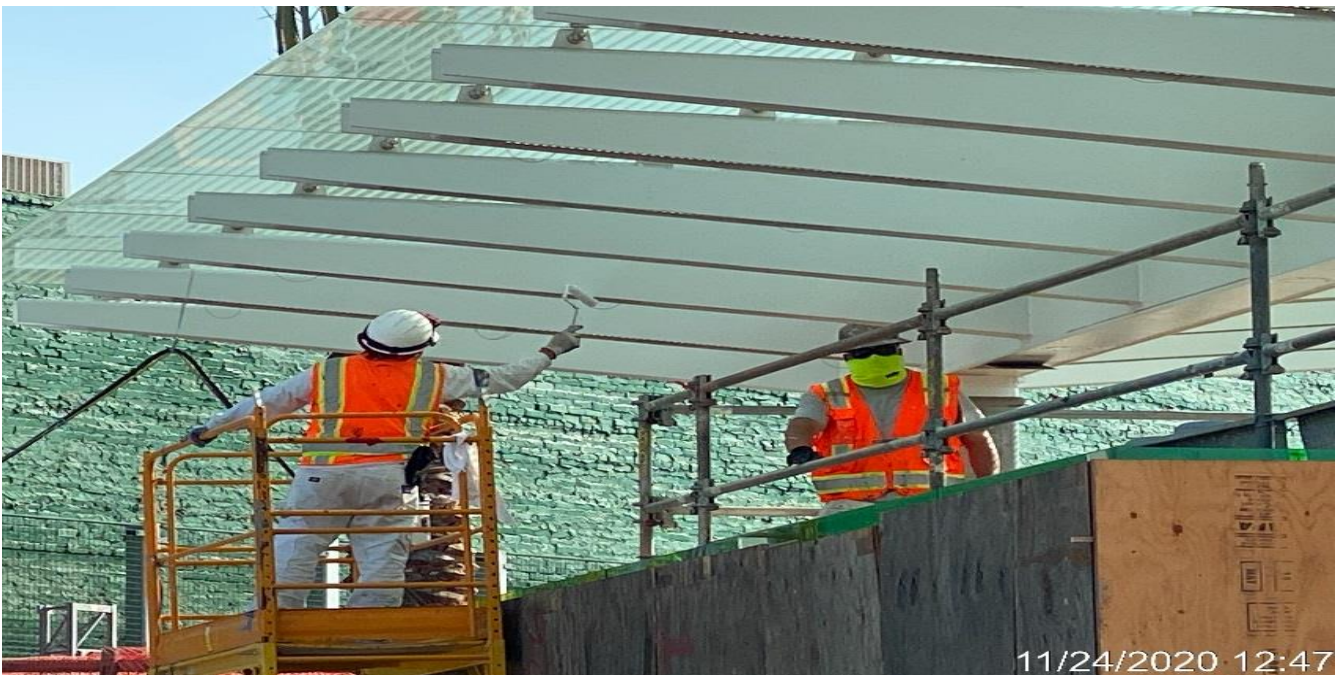
LEIMERT PARK STATION – Applying finish paint to the main entrance canopy outriggers at the plaza.
