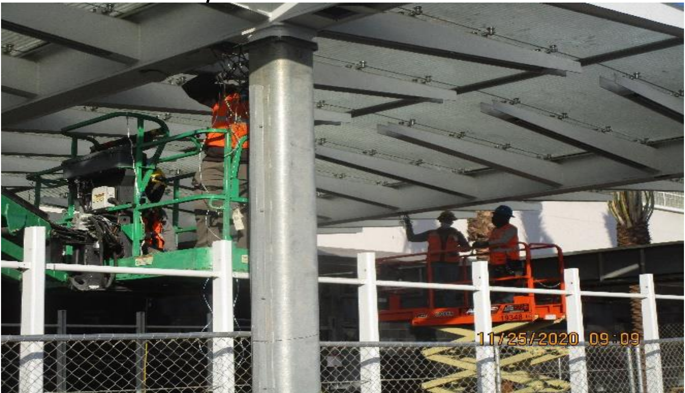
MLK STATION – MLK Plaza, entrance canopy continued terminating #12 normal & emergency lighting (hot, neutral ground).
