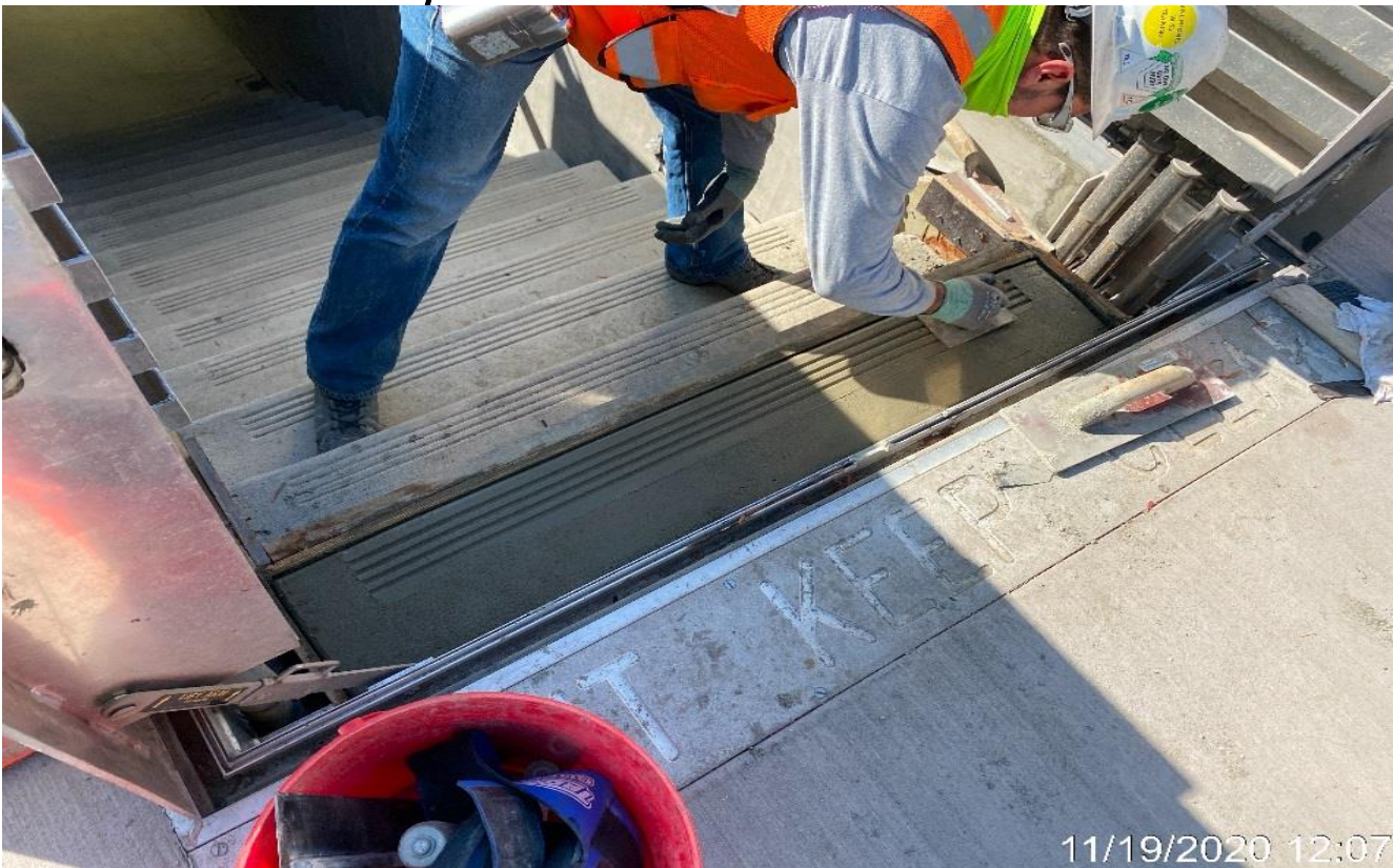
LEIMERT PARK STATION – Placing concrete for the top step of Emergency Exit Stair 1 at the plaza.
