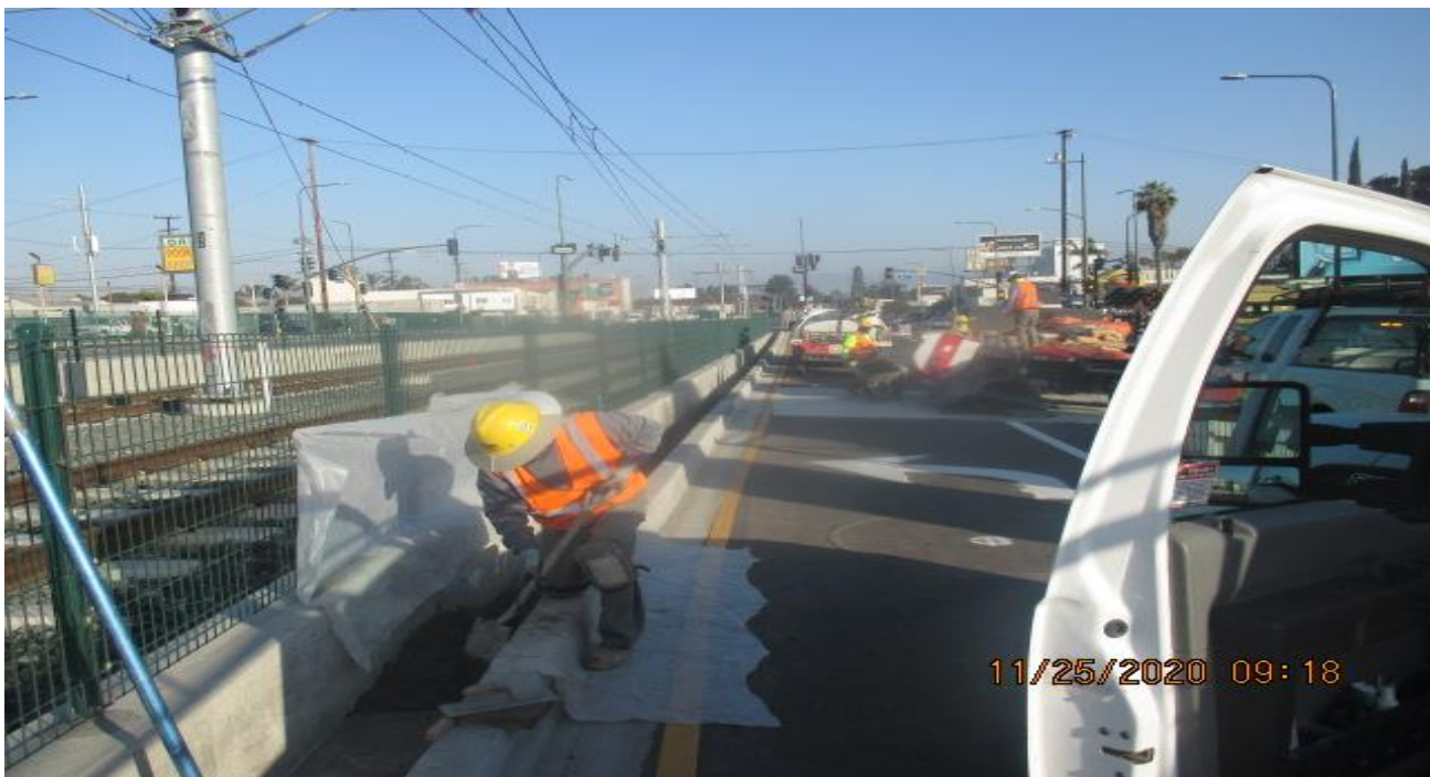
PARK MESA – Continue placing mortar on the northbound median curb on Crenshaw Blvd from 50th St to 48th St.
