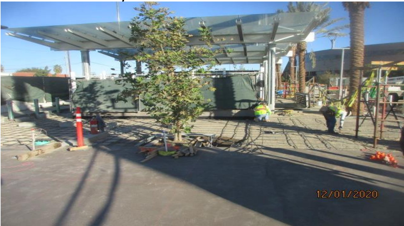
EXPO STATION – Continue building formwork and placing rebar for the architectural topping slab at the center section of the plaza.
