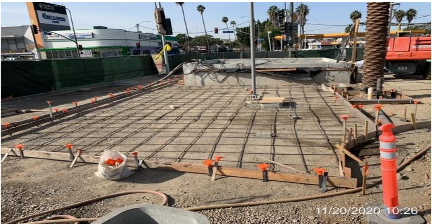
EXPO STATION – Dean Visosky tying rebar and setting formwork for concrete slab.
