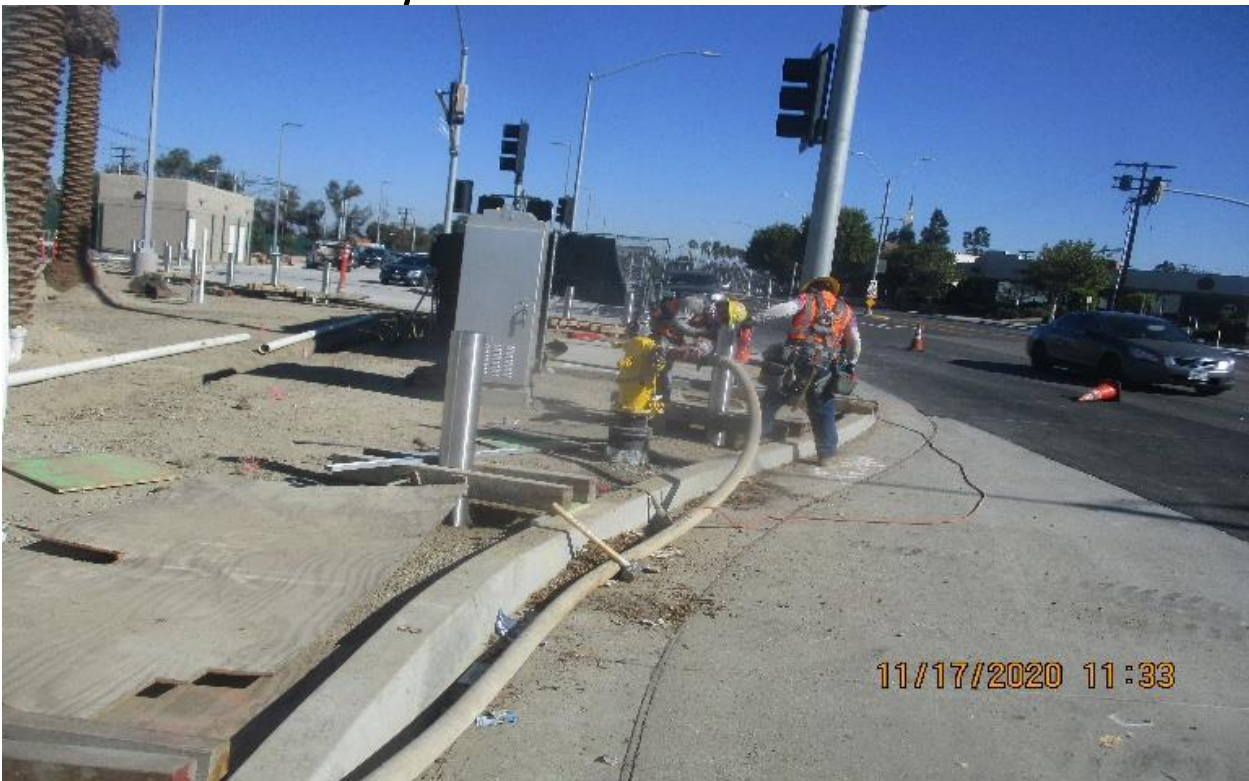
La Brea – WSCC Set and place concrete for bollards at La Brea park and ride exit.
