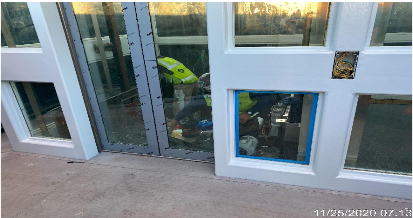
LEIMERT PARK STATION – Caulking and sealing glass panels for Elevators 1&2 at the plaza.
