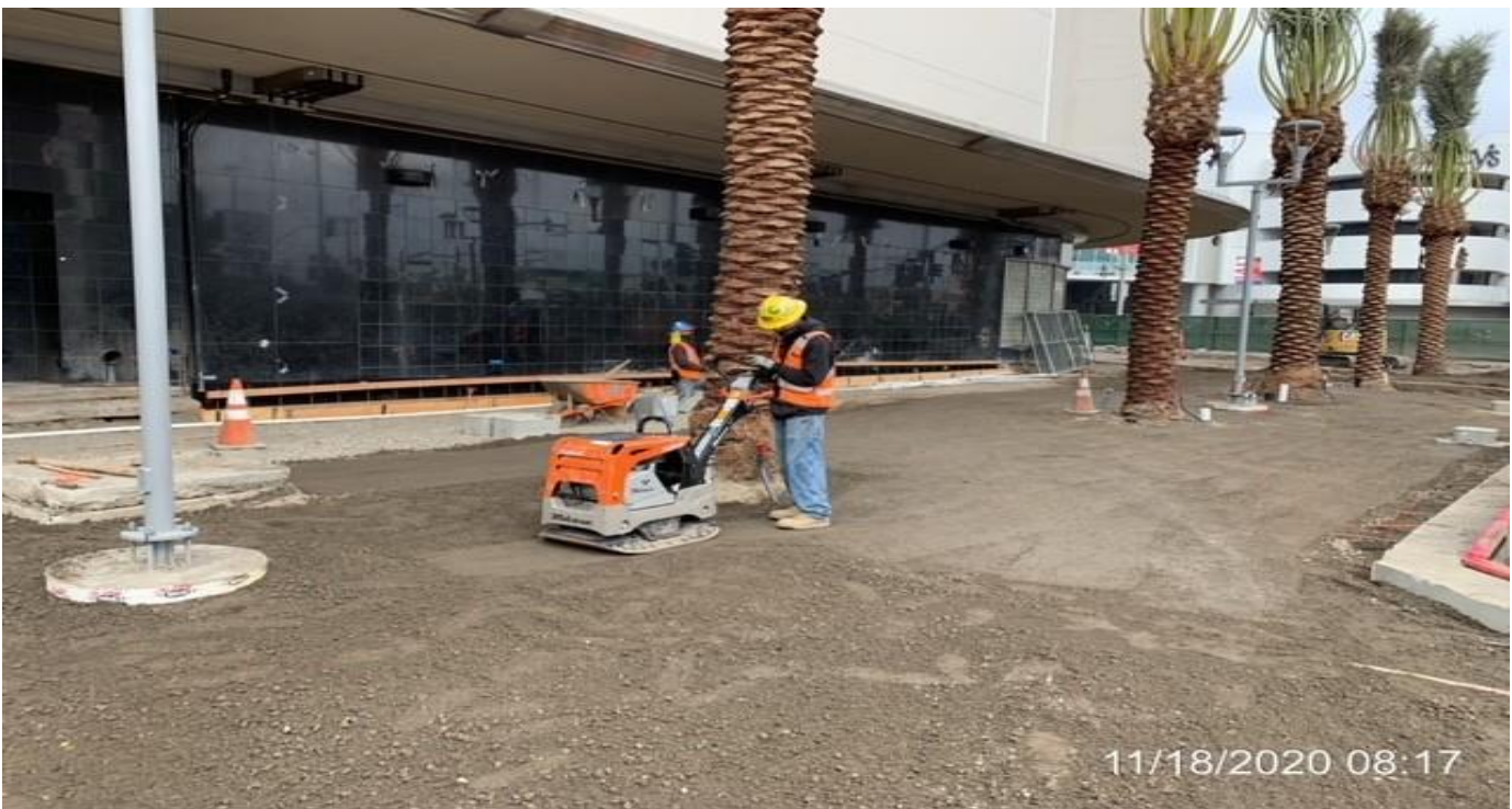
MLK STATION – Continue laying base and compacting the north end area of the plaza.
