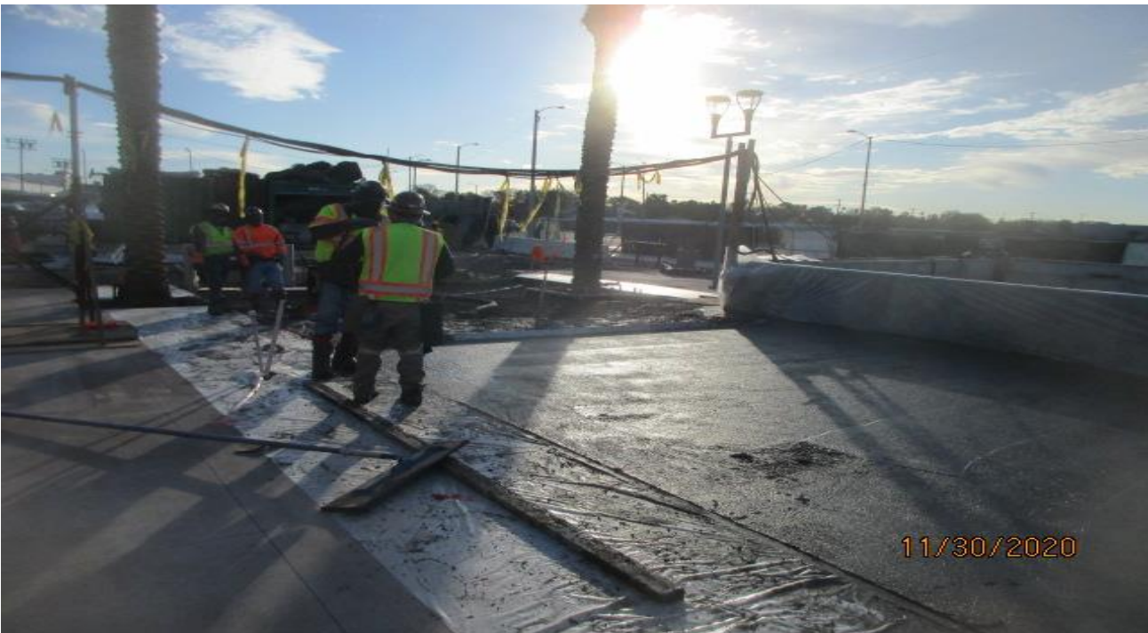
EXPO STATION – Continue building formwork and placing rebar for the architectural topping slab at the south end section of the plaza.
