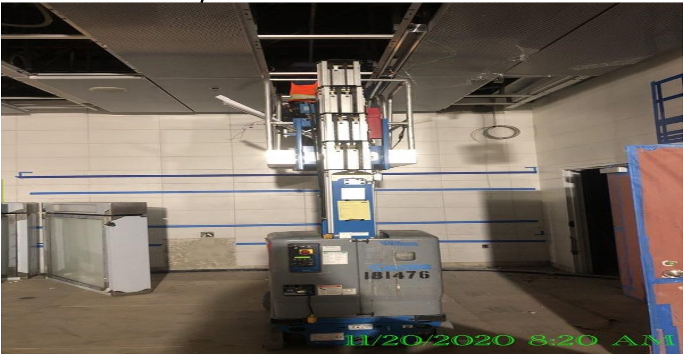
MLK STATION – Installing LED light fixtures to the ceilings of the Paid Area at the concourse.
