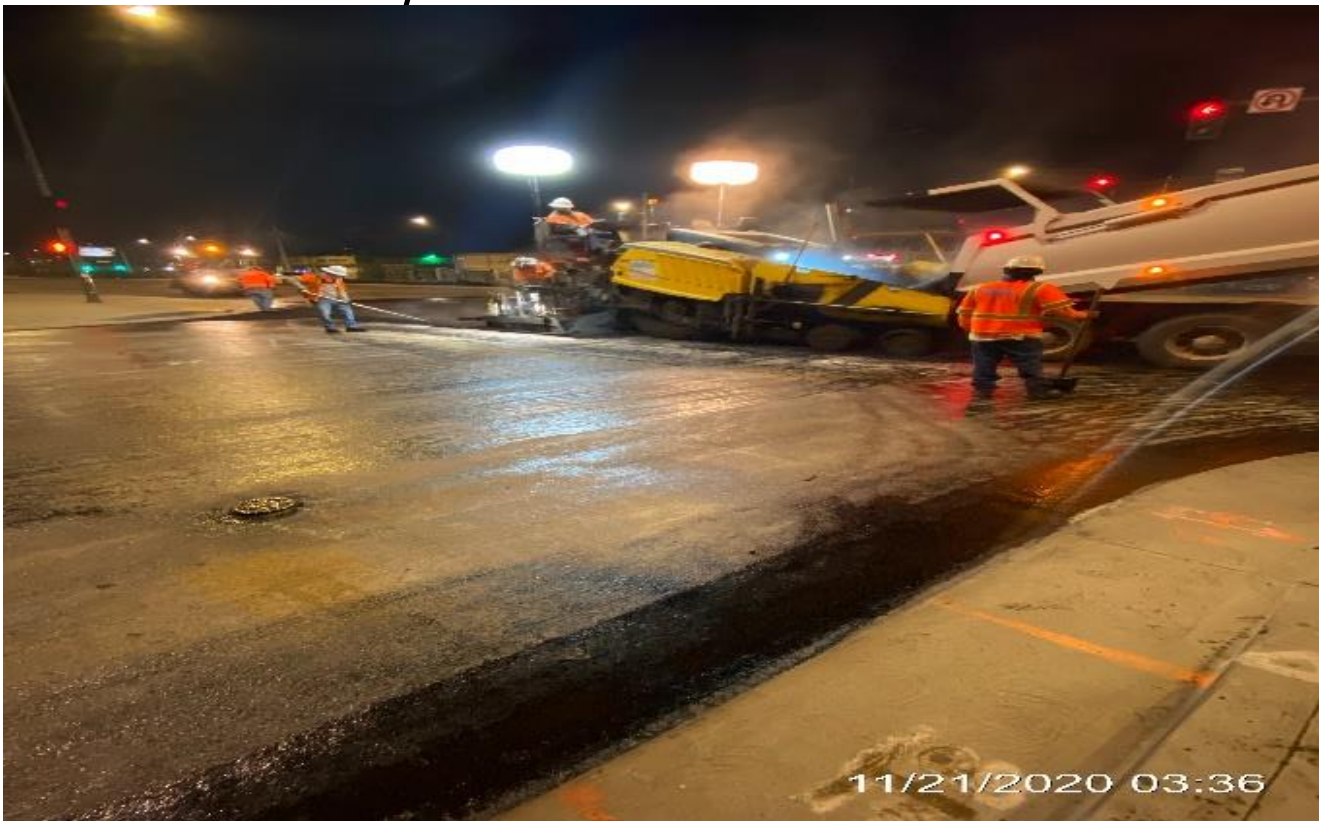
PARK MESA – Grinding and paving the north and southbound lanes at Crenshaw Blvd and 57th St
