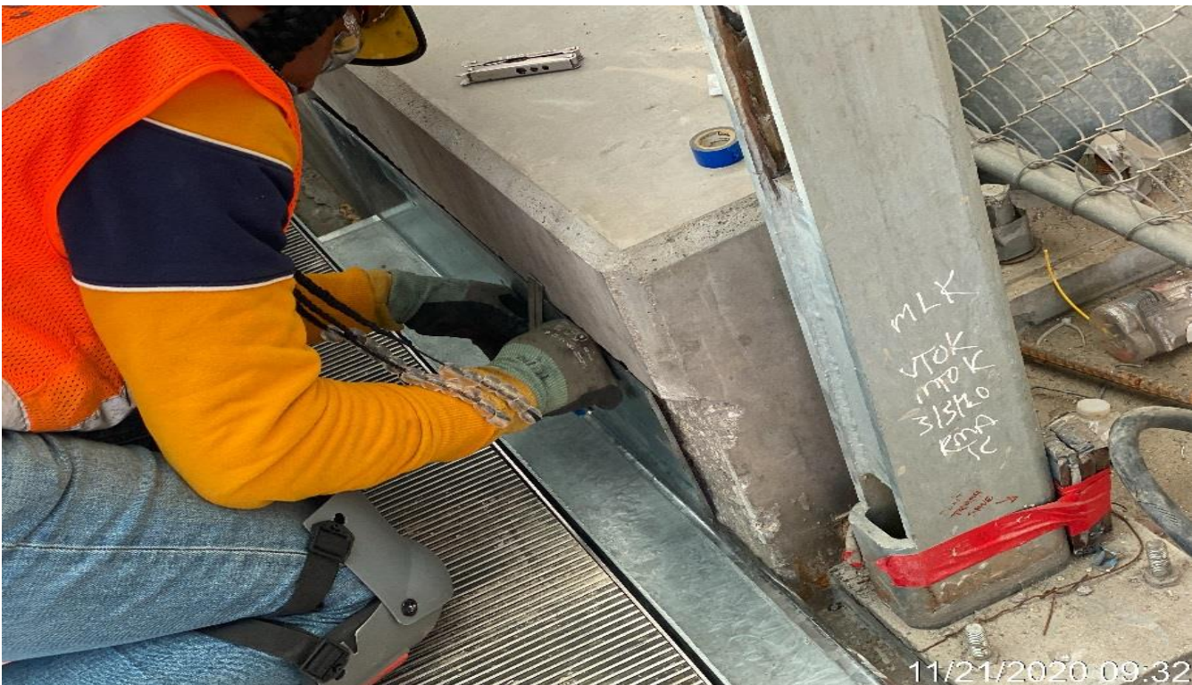
MLK STATION – Installing steel mud pans to the edges of Escalators 1&2 at the main entrance of the plaza.
