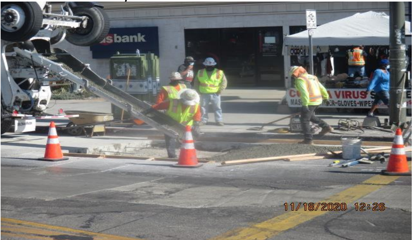
PARK MESA – Placing rebar and concrete for road section on the northeast corner of Crenshaw Blvd and Slauson Ave.
