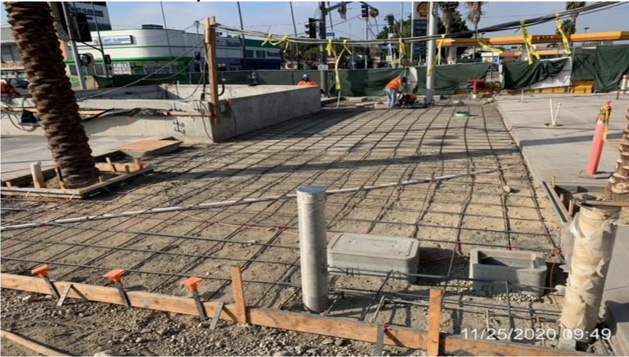
EXPO STATION SITE – Continue building formwork and placing rebar for the architectural topping slab at the south end section of the plaza.
