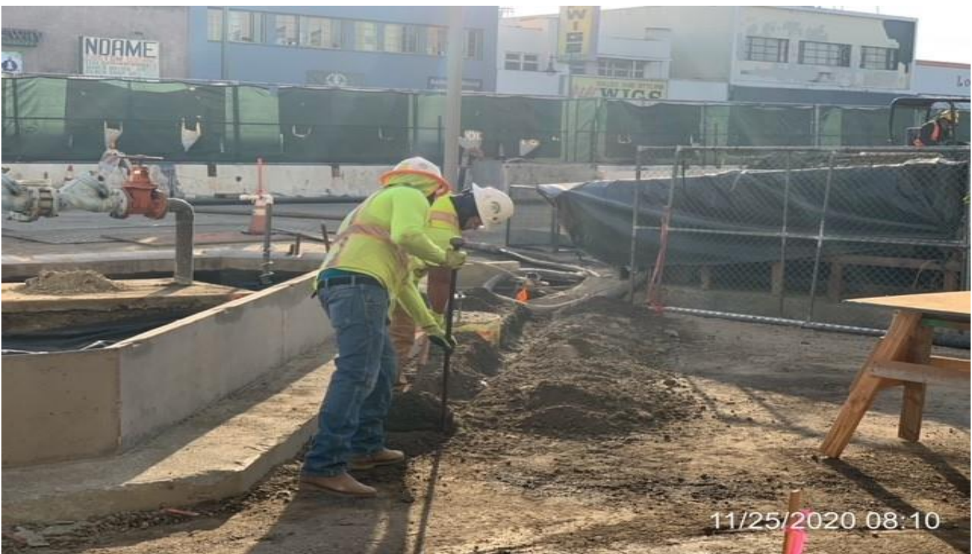
MLK STATION – Digging for backflow irrigation for the North planter wall at the plaza.
