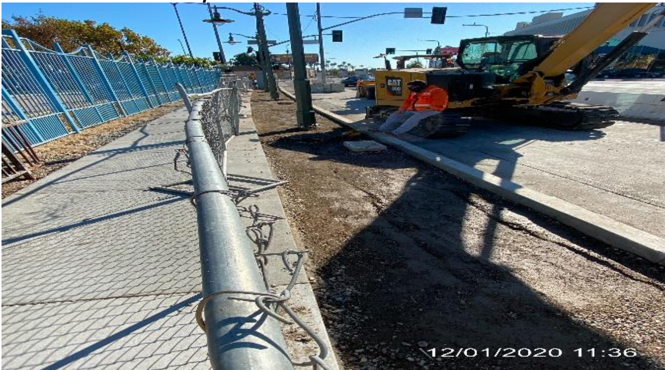
LEIMERT PARK STATION – Continue fine grading and compacting sidewalk on northbound Crenshaw Blvd between Vernon Ave and 43rd Pl.
