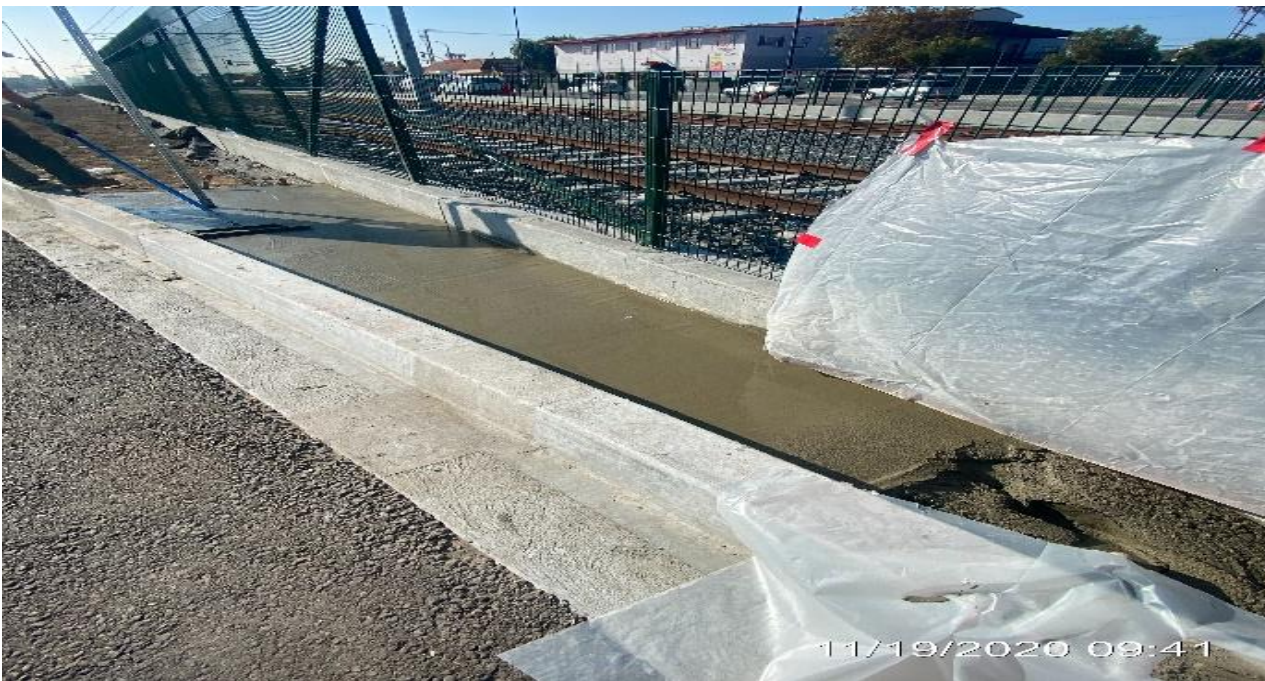
PARK MESA – Placing mortar on the northbound median curb on Crenshaw Blvd from Slauson Ave and 57th St.
