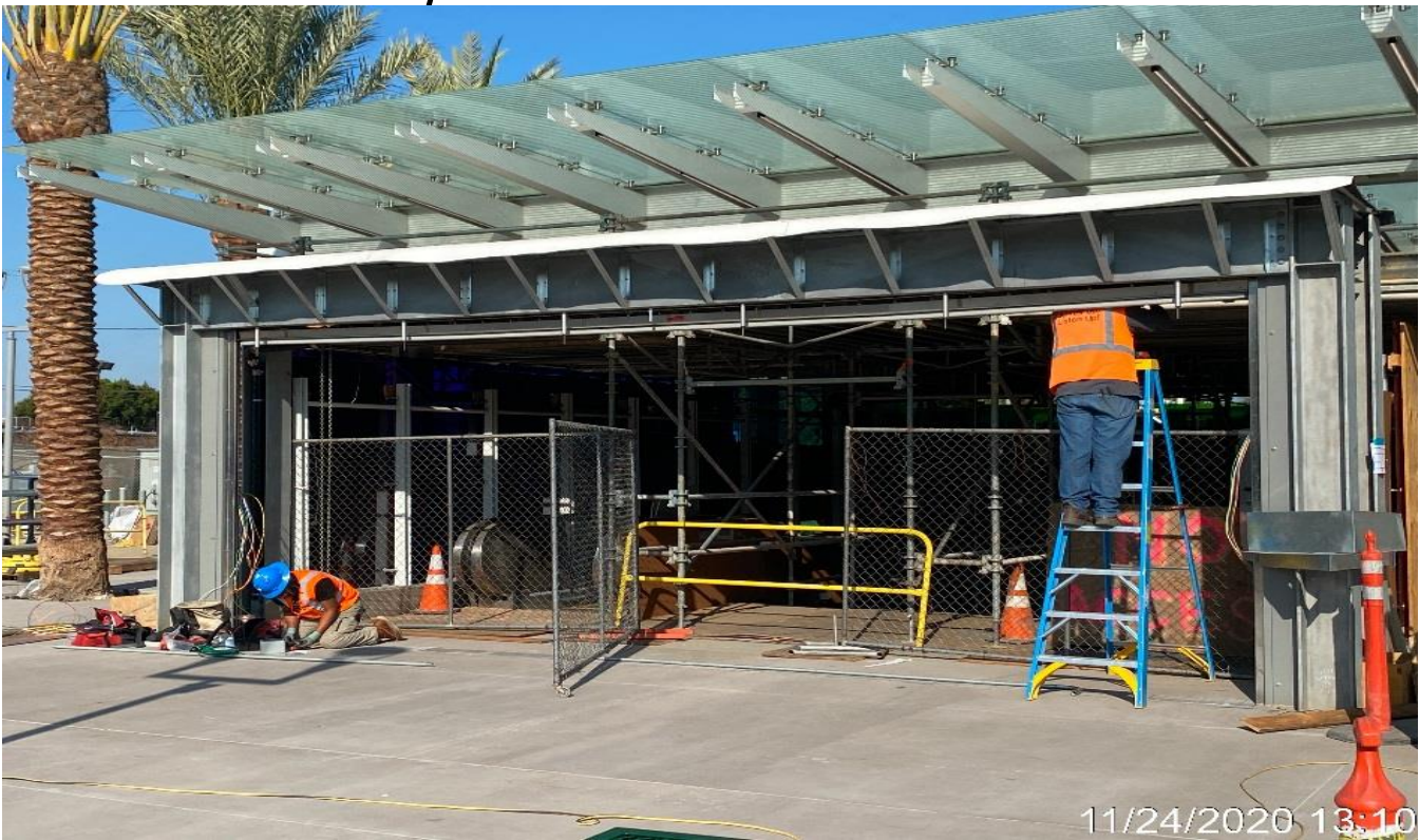
LEIMERT PARK STATION – Wiring up the main entrance roll-up gate at the plaza.
