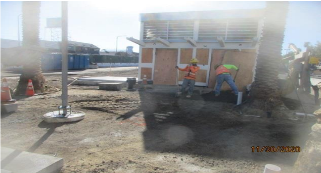
MLK STATION – Continue laying base and compacting the south end area of the plaza.
