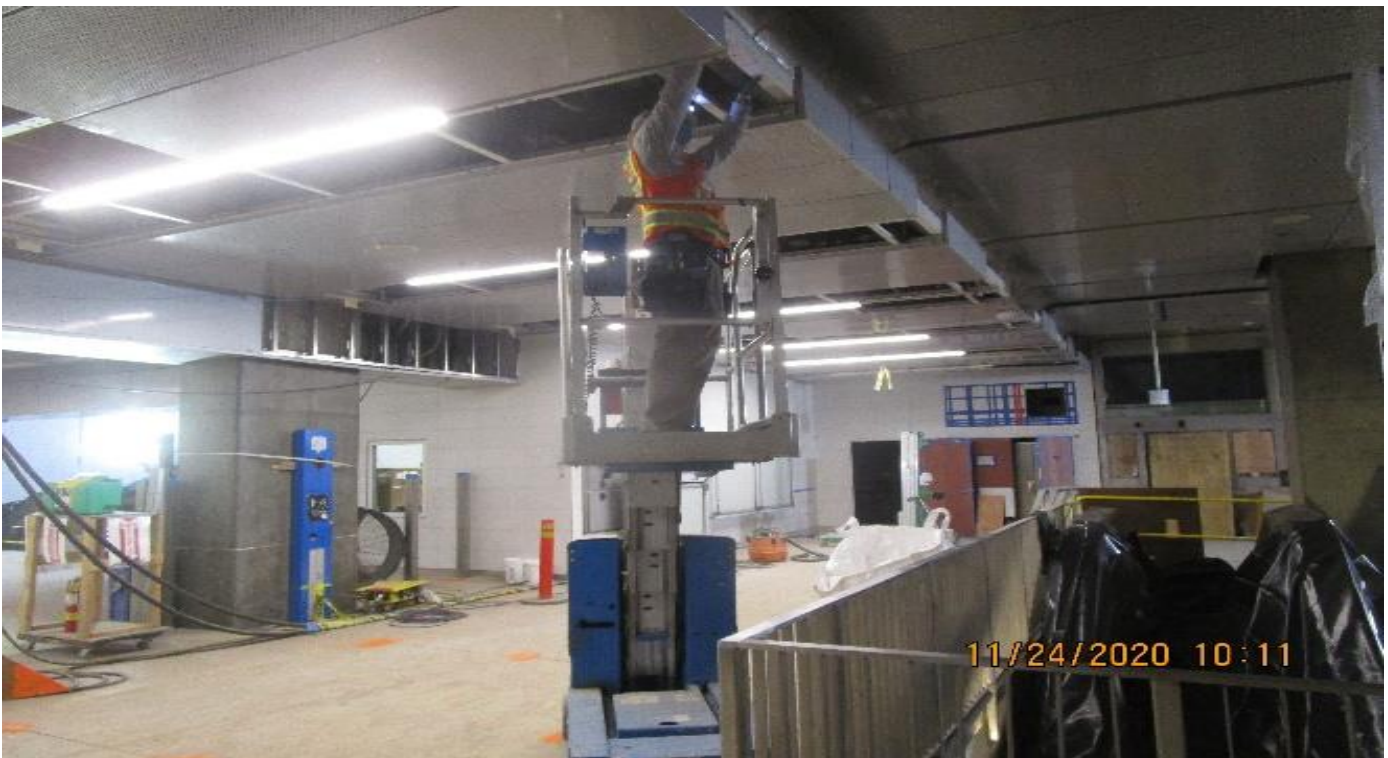
MLK STATION – Continue installing LED light fixtures to the ceilings of the Paid Area at the concourse.
