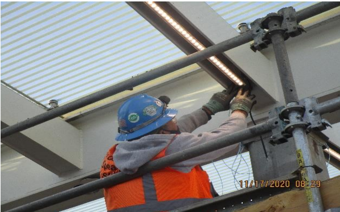
UG3 – Vernon Plaza, Entrance canopy BOCA emergency & normal LED light fixtures begin trouble shooting.
