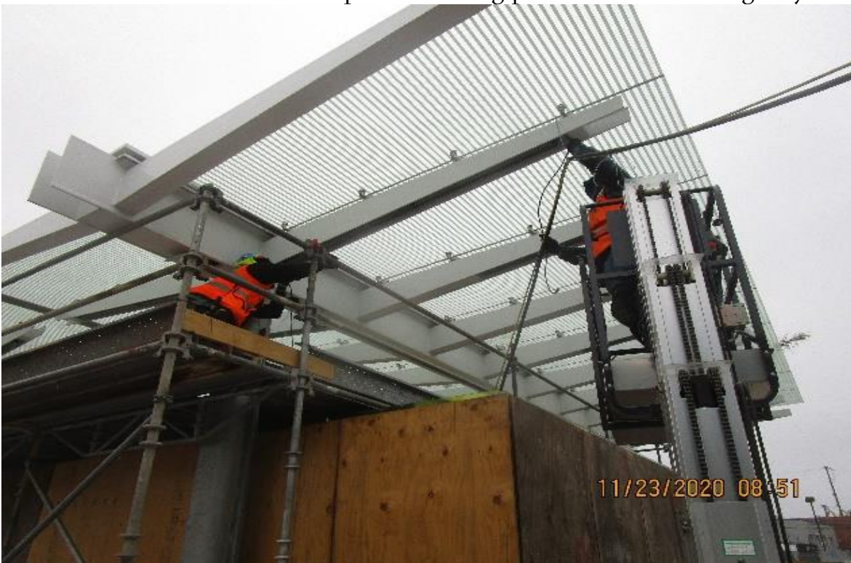
UG3 – Vernon Plaza, Entrance canopy BOCA emergency & normal LED light fixtures begin trouble shooting.
