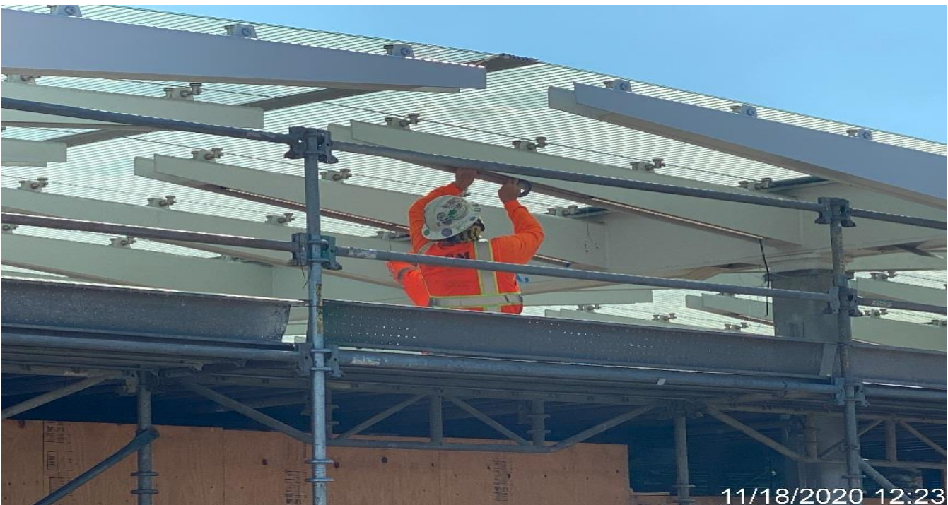
LEIMERT PARK STATION – Continue installing BOCA light fixtures to the main entrance canopy outriggers at the plaza.
