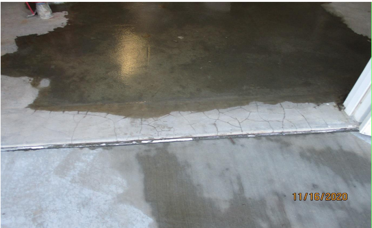
AVIATION/CENTURY- Cracking concrete at the Aviation Station service building door flooring.
