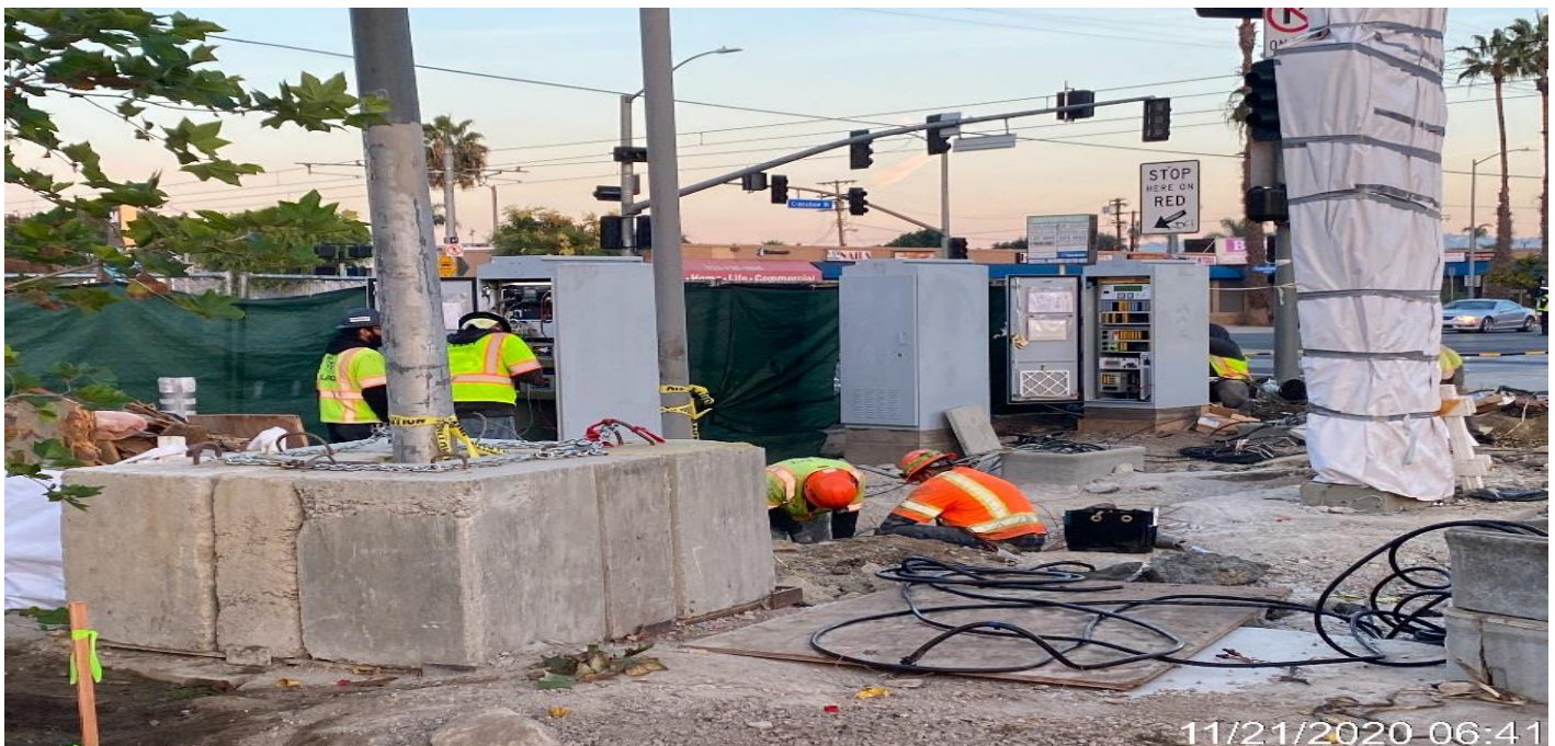
EXPO STATION – Continue installing controller cabinets at the northwest corner area of the plaza and connecting fiber optic conduits to the controller cabinets.
