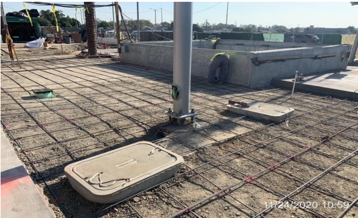
EXPO STATION – Dean Visosky tying rebar for 3 shades of grey concrete slab.
