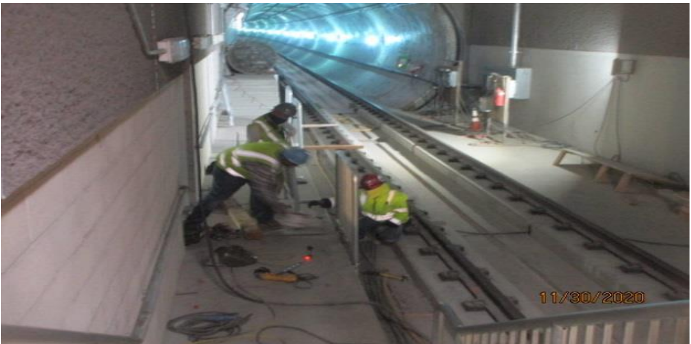
MLK STATION – Installing guardrails at the North and South Back of House along both the north and southbound side of the platform.
