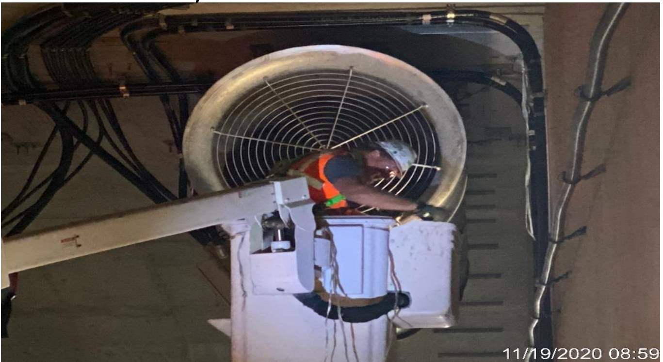
LEIMERT PARK STATION – Performed inspections of all the tunnel booster fans in preparation for start-up/energization.
