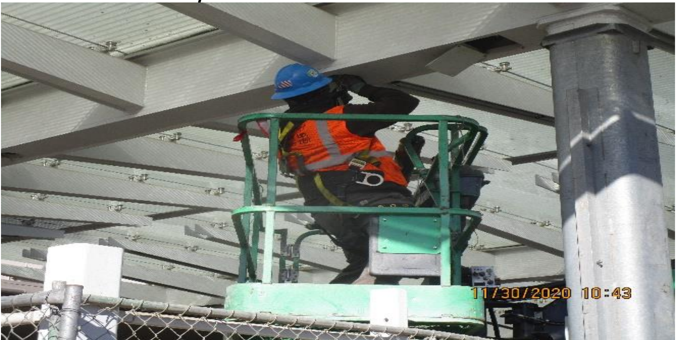
MLK STATION – Continue BOCA light fixture installation to the main entrance canopy outriggers at the plaza.
