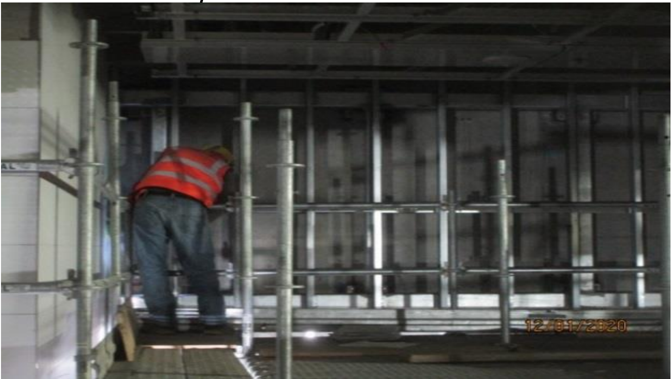
EXPO STATION – Continue installing cement board sheet to the furred out wall for the Mosaic Art Wall at the concourse.
