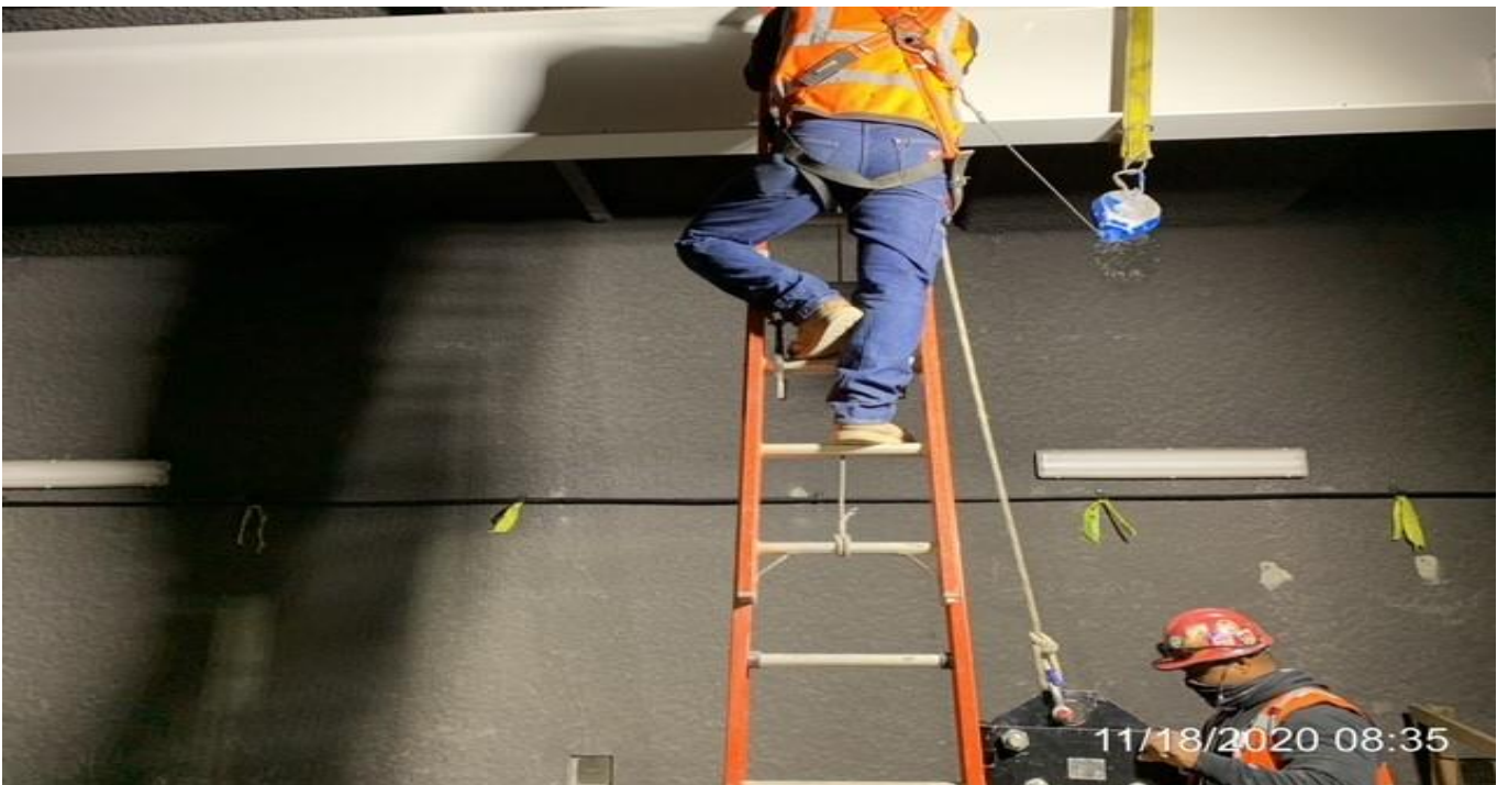
MLK STATION – Installing trolley beams to the walls inside the Tunnel Vent/OTE Plenum South C-101 at the concourse.
