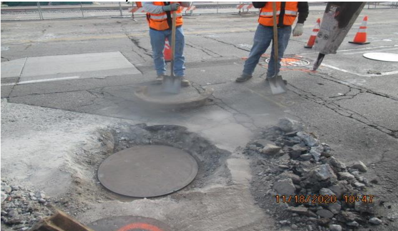
PARK MESA – Removing rings and access covers of sewer maintenance holes and placing protective plates prior to grind and overlay on southbound Crenshaw Blvd and 59th St.
