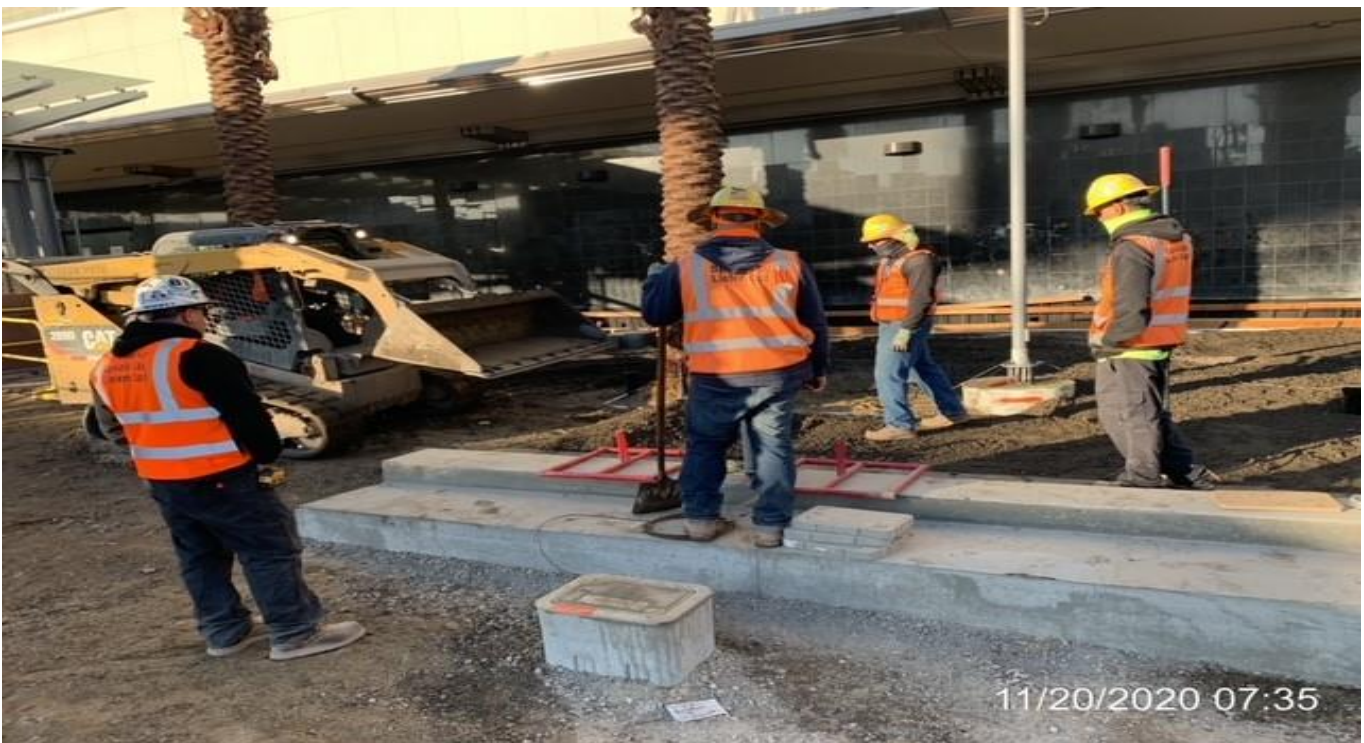
MLK STATION – Continue laying base and compacting the north end area of the plaza.
