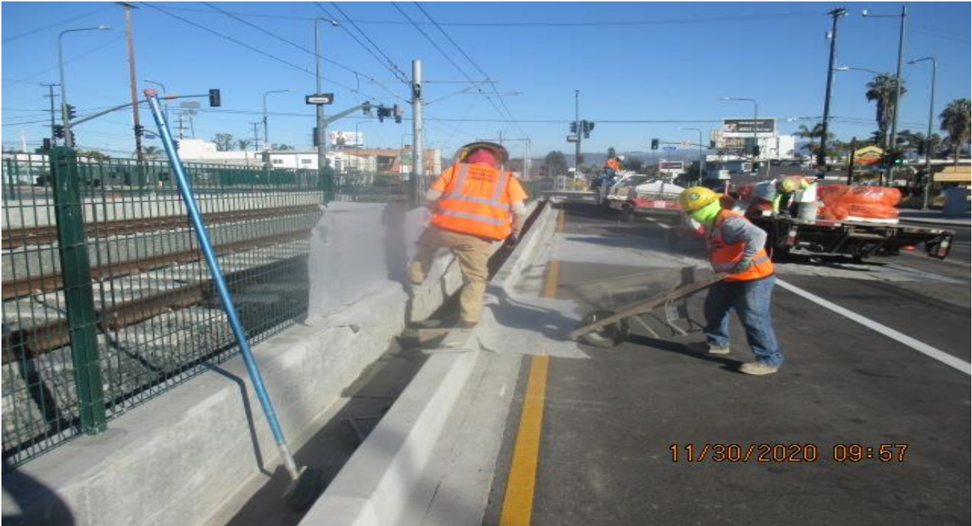
PARK MESA – Continue placing mortar on the northbound median curb on Crenshaw Blvd from 50th St to 48th St.
