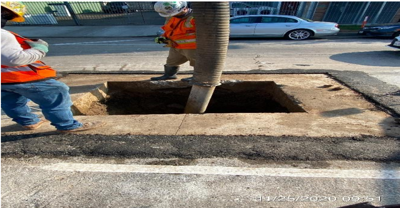
PARK MESA – Potholing for the removal of an existing overhead sign foundation on northbound Crenshaw Blvd and 48th St.
