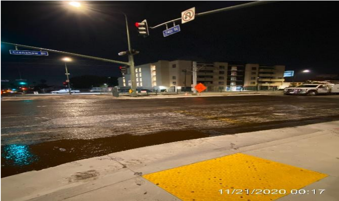
PARK MESA – Grinding and paving the north and southbound lanes at Crenshaw Blvd and 54th St.
