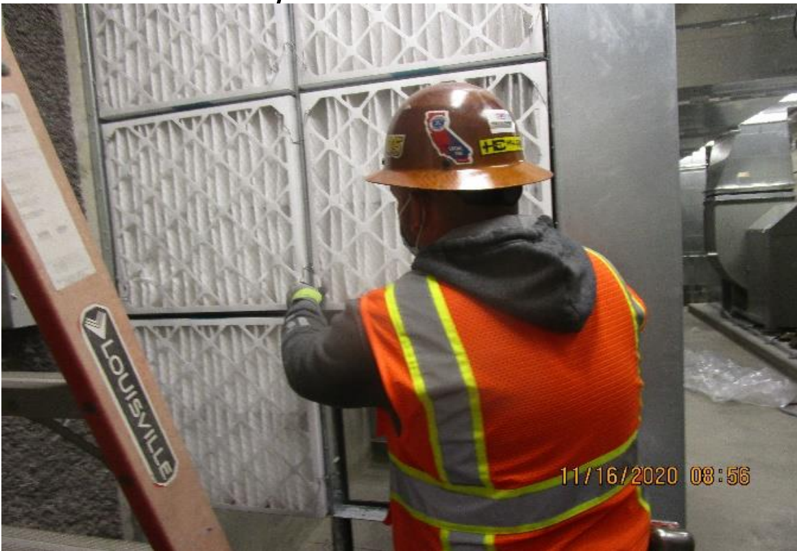
UG3 – Vernon, Mechanical room (N) C135, begin installing Flanders 40 Merv-8 pleated filters at F-6-1 & filter media.
