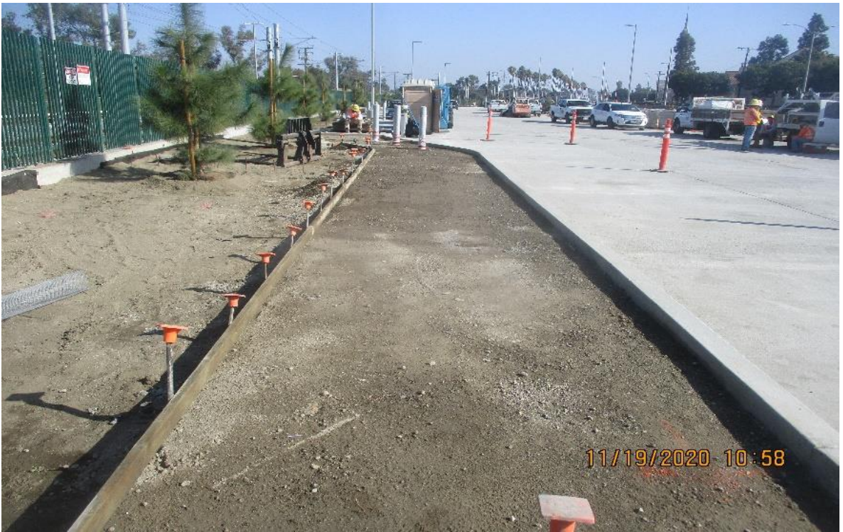
La Brea – WSCC Form and place SWK concrete at La Brea Park and ride.
