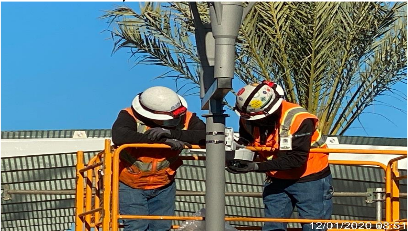
LEIMERT PARK STATION – Installing CCTV cameras to the pedestrian street light poles at the plaza.
