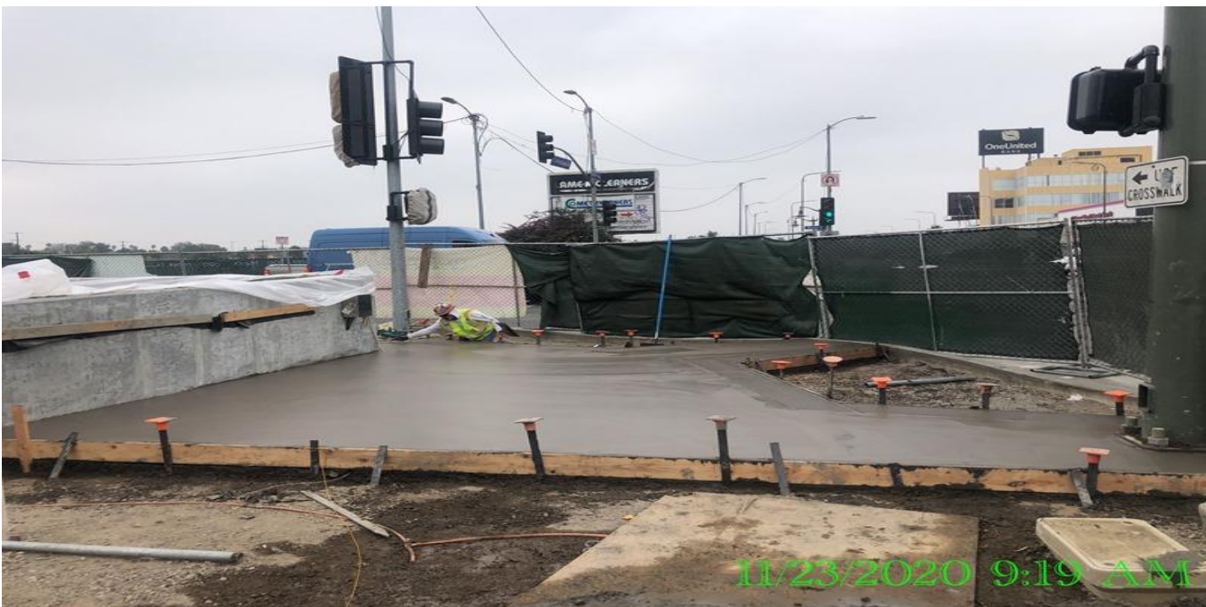
EXPO STATION– Placing concrete for the architectural topping slab at the south end section of the plaza.
