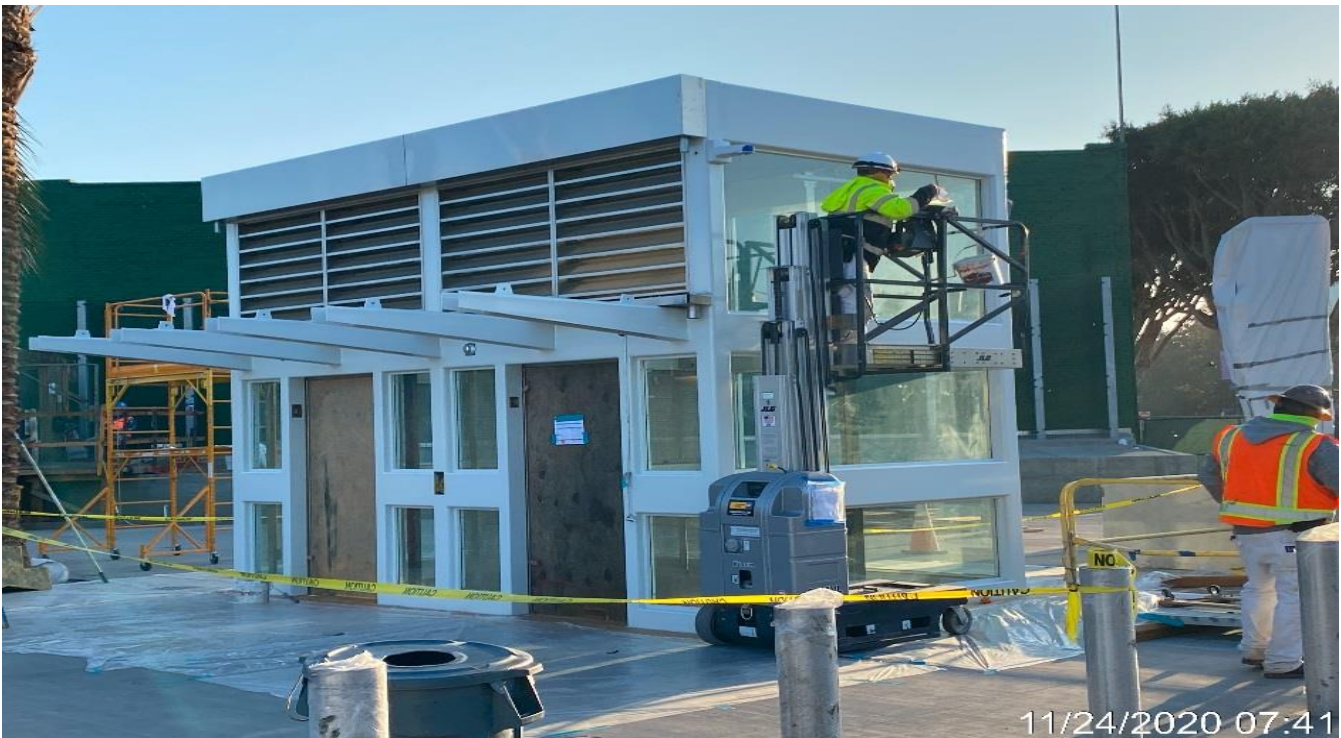
LEIMERT PARK STATION – Applying finish paint to the outriggers of Elevators 1&2 at the plaza.
