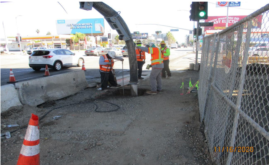
AVIATION/CENTURY- Potholing for the proposed storm drain catch basin on the SW corner of Aviation and Century.
