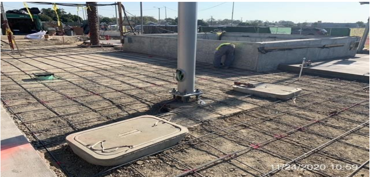
EXPO STATION SITE – Continue building formwork and placing rebar for the architectural topping slab at the south end section of the plaza.
