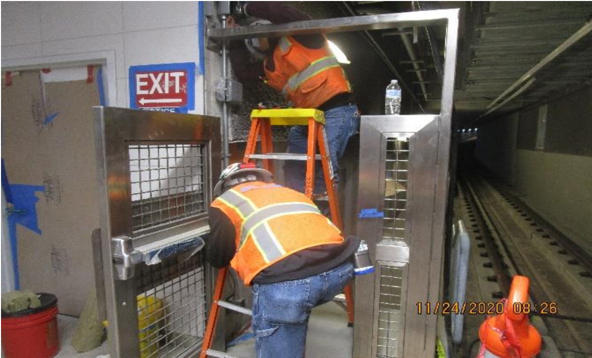
UG3 – Vernon Platform, north & southbound end gates resume rough in of SCADA security door strobes & door contacts.
