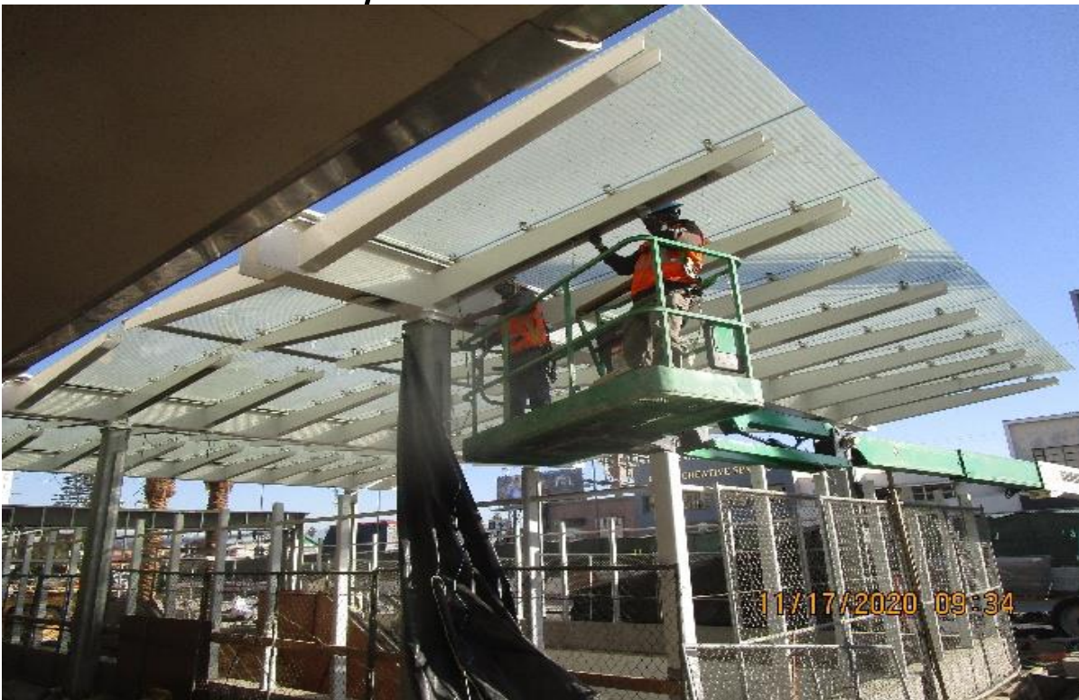
MLK STATION – MLK (S) Plaza, Entrance canopy outriggers begin installing BOCA emergency & normal lighting fixtures.
