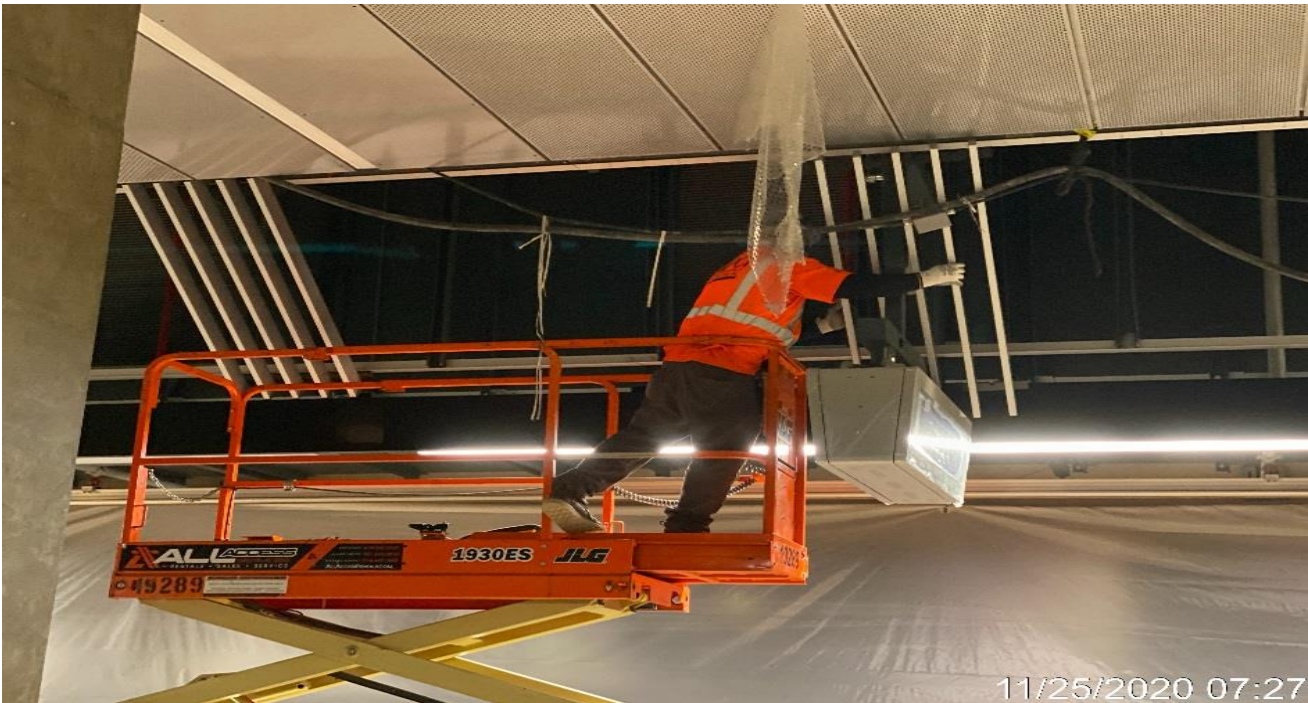
LEIMERT PARK STATION – Resume diagonal screen panel installation along the north and southbound side of the platform.
