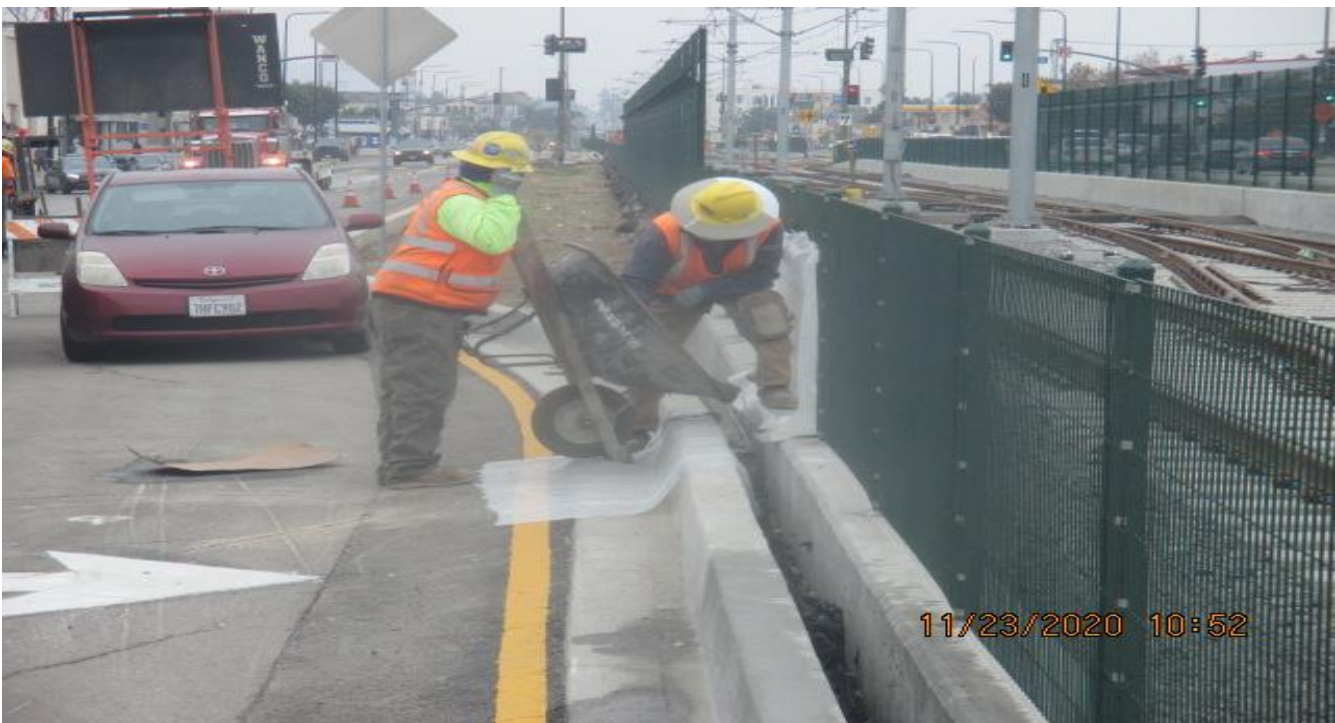
PARK MESA – Continue placing mortar on the northbound median curb on Crenshaw Blvd from 57th St to 54th St.
