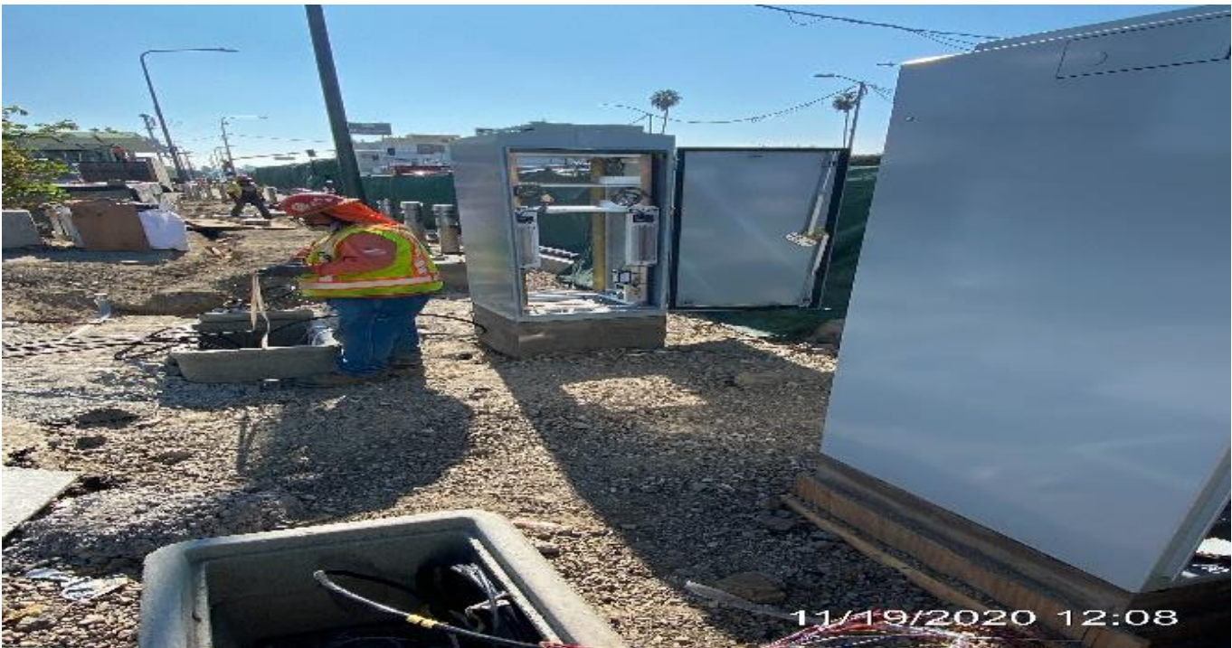
EXPO STATION– Installing controller cabinets at the northwest corner area of the plaza.
