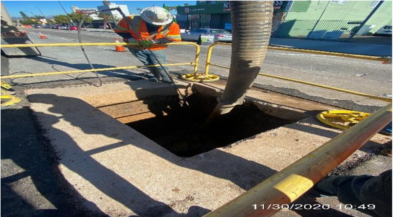
PARK MESA – Continue potholing for the removal of an existing overhead sign foundation on northbound Crenshaw Blvd and 48th St.
