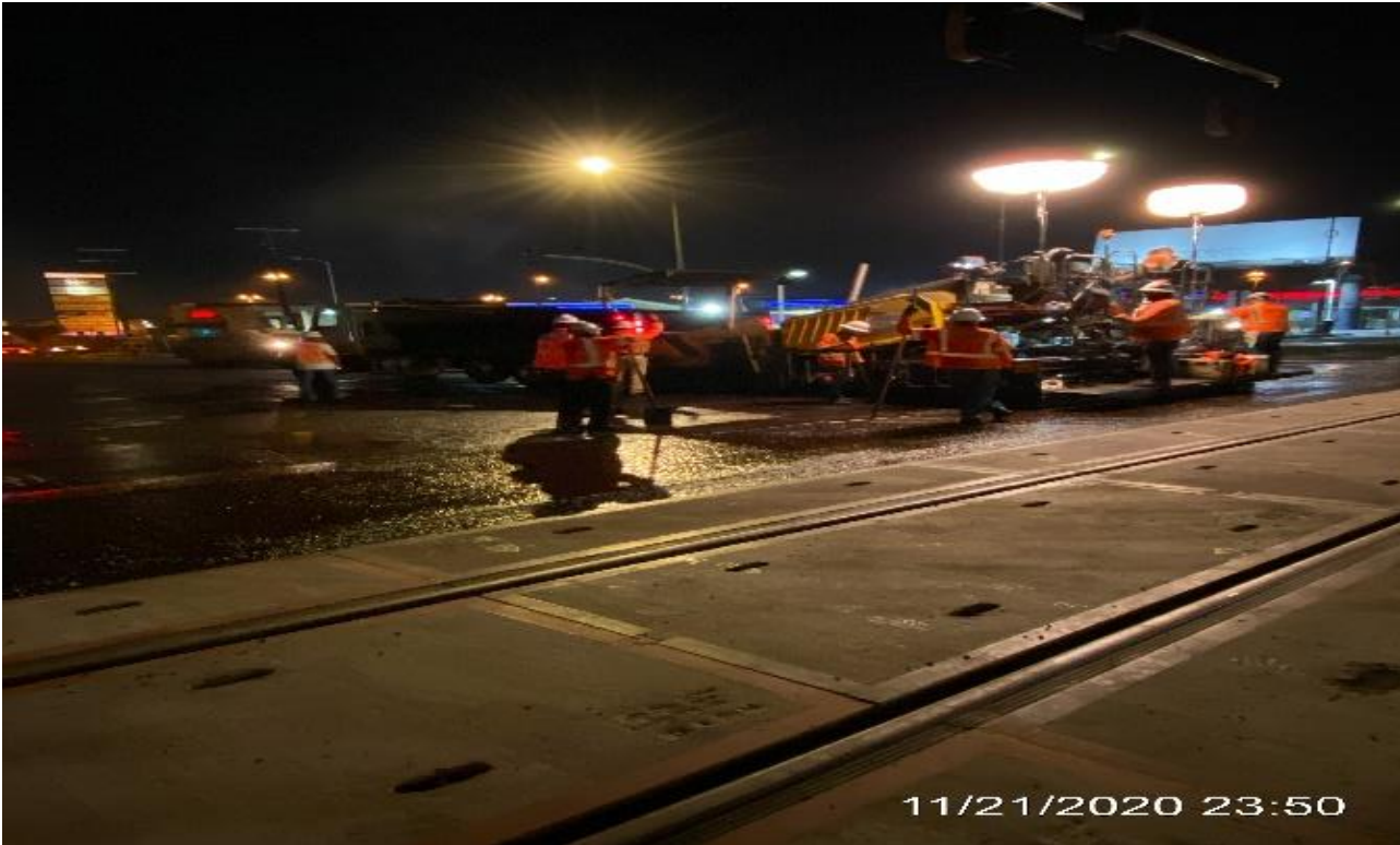
PARK MESA – Grinding and paving the north and southbound lanes at Crenshaw Blvd and Slauson Ave.
