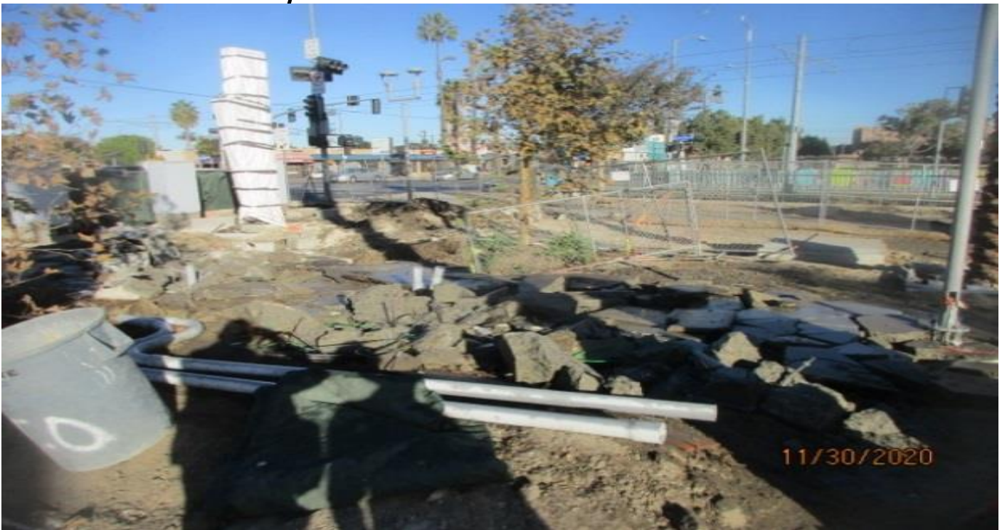
EXPO STATION – Removing abandoned controller cabinet foundation at northwest corner area of the plaza.
