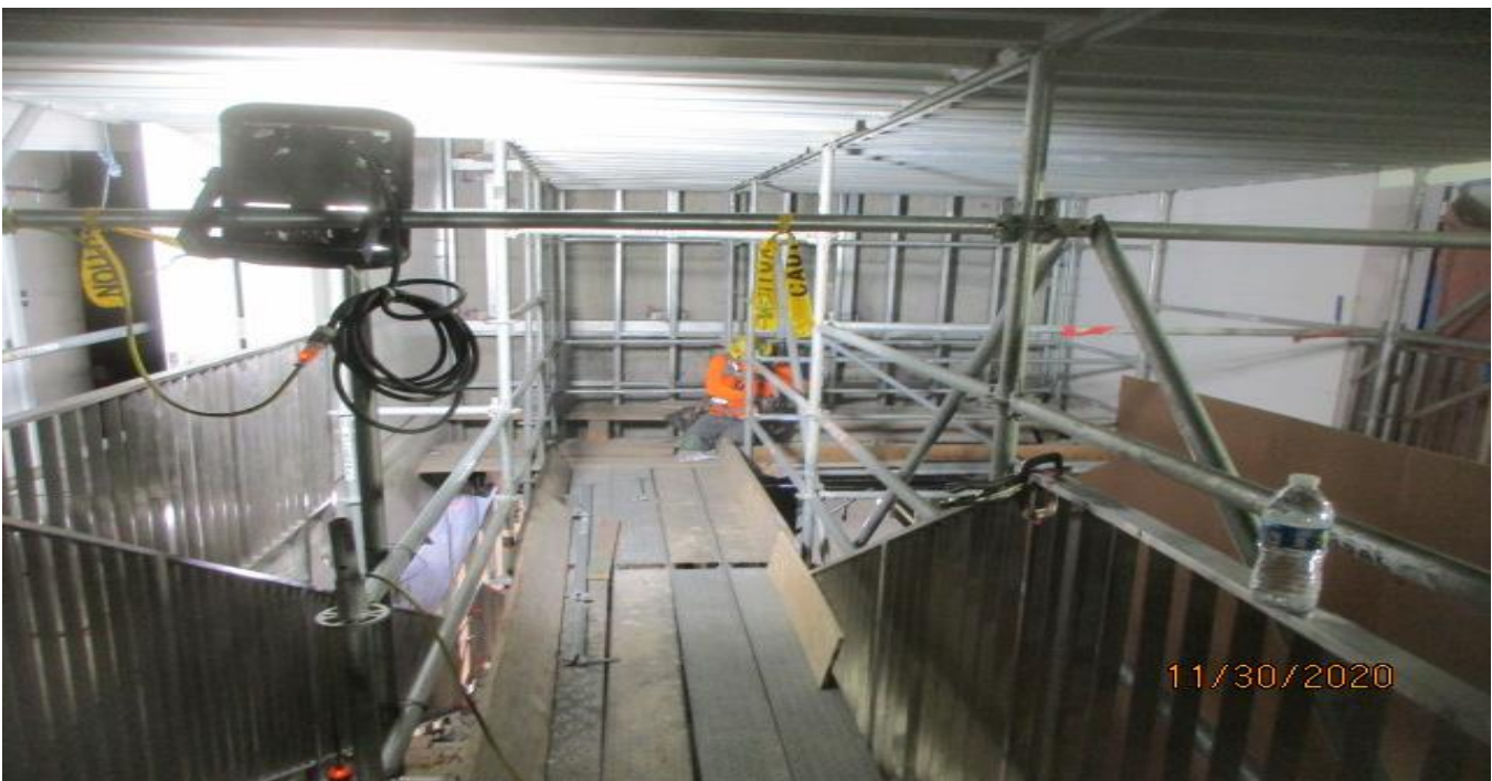
EXPO STATION – Installing cement board sheet to the furred out wall for the Mosaic Art Wall at the concourse.
