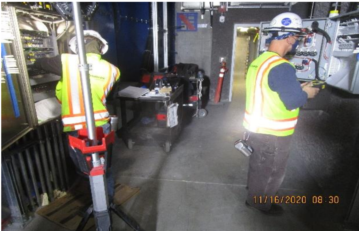
UG3 – Vernon, EM Fan room (S) C102 EVF-6-302, LCS continued terminating #14 XHHW-2, control wiring.
