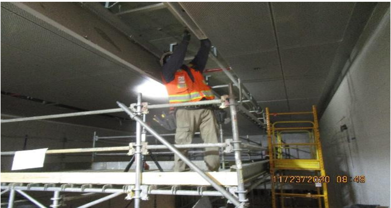
LEIMERT PARK STATION – Installing LED light fixtures to the ceiling of the intermediate landing.
