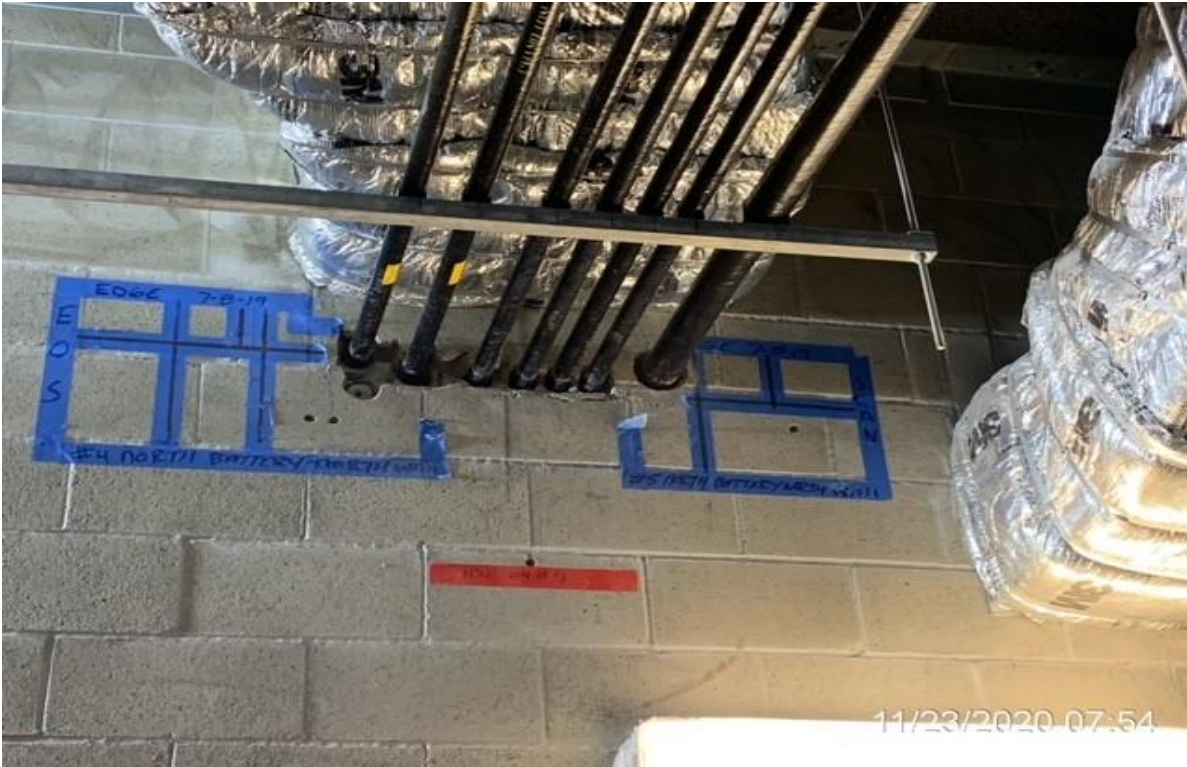
UG3 – VERNON – Bielski fire proof caulking penetrations at emergency fan room north.
