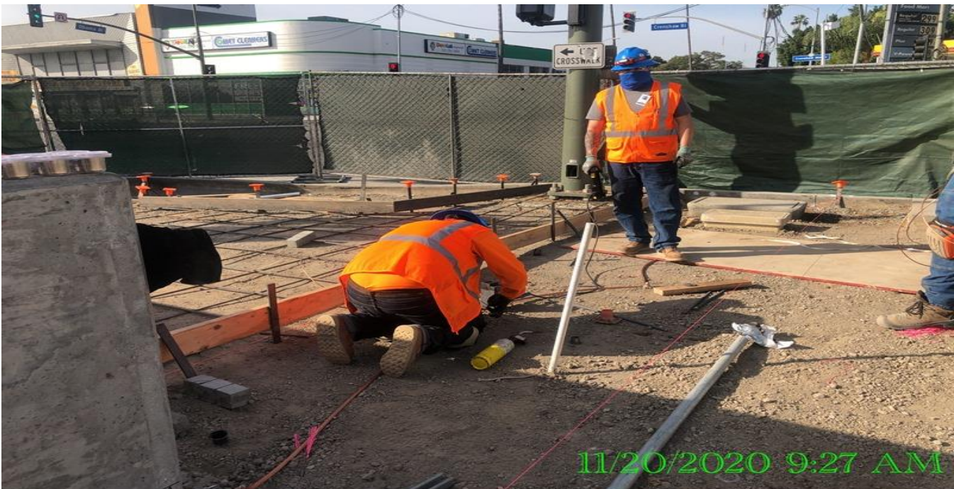
EXPO STATION – Installing ground grid system at the southwest section of the plaza.
