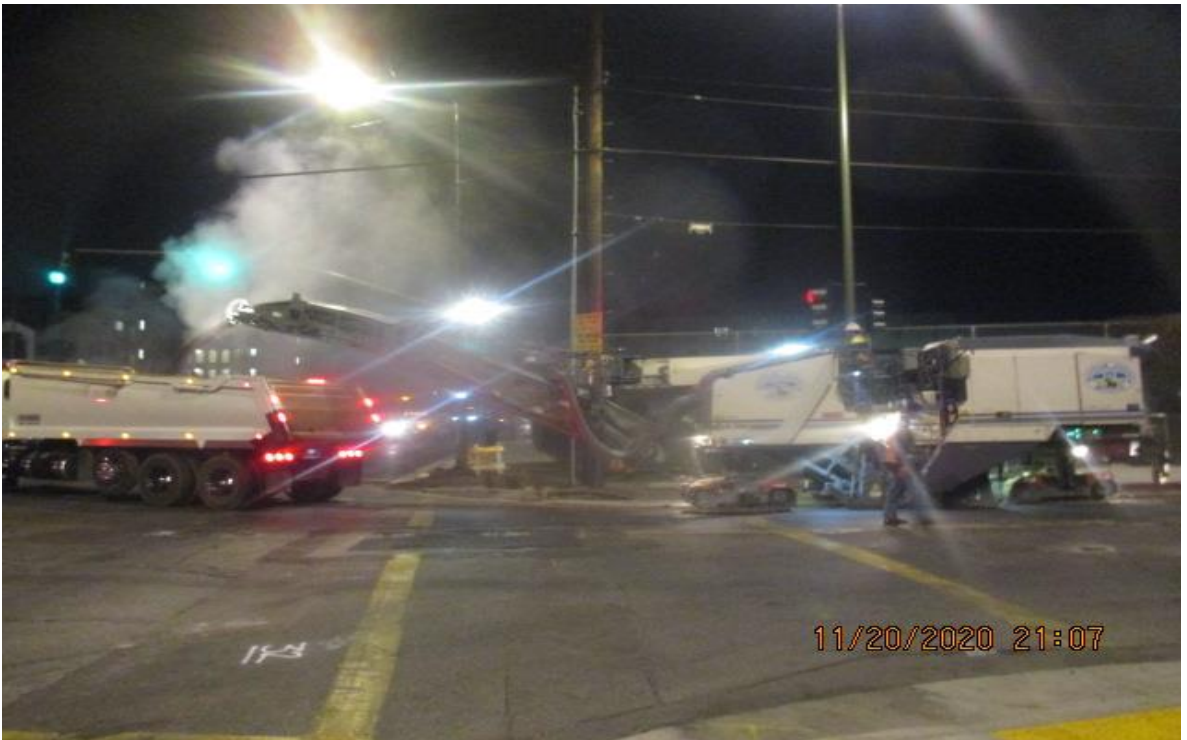
PARK MESA – Grinding and paving the north and southbound lanes at Crenshaw Blvd and 60th St..
