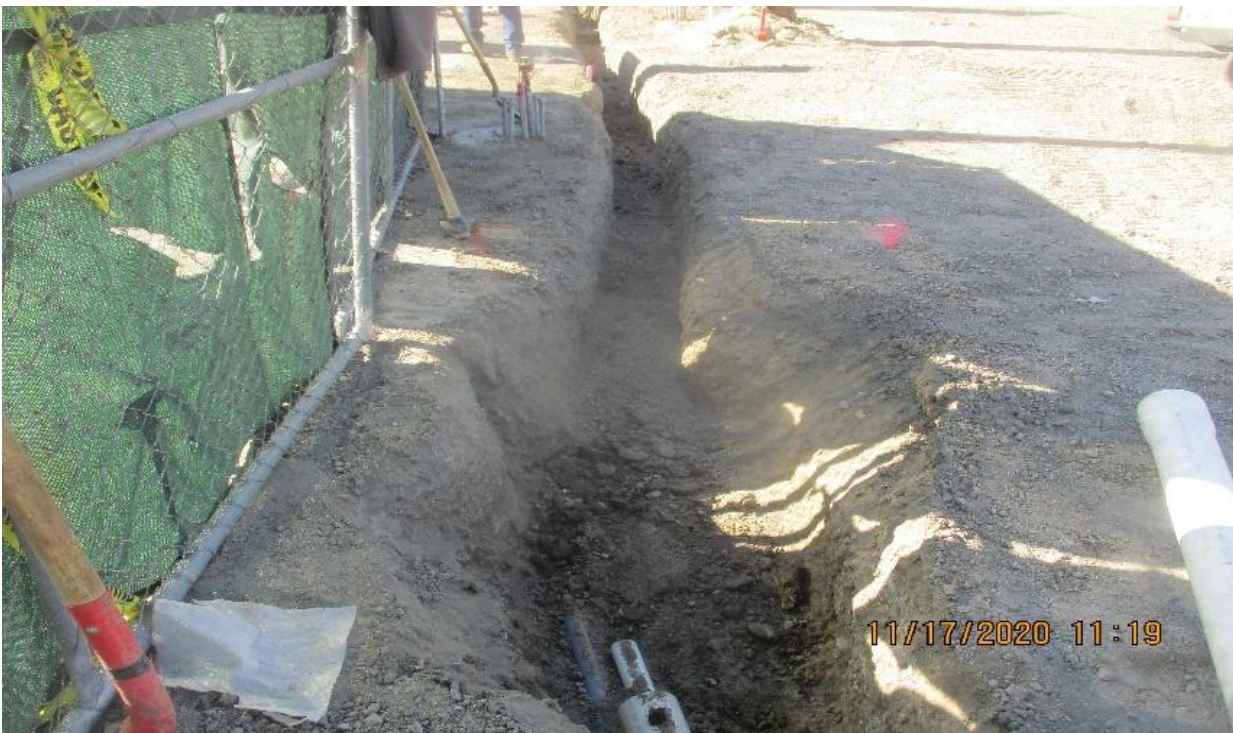
La Brea – Marina Excavate trench for main line water at La Brea Plaza.
