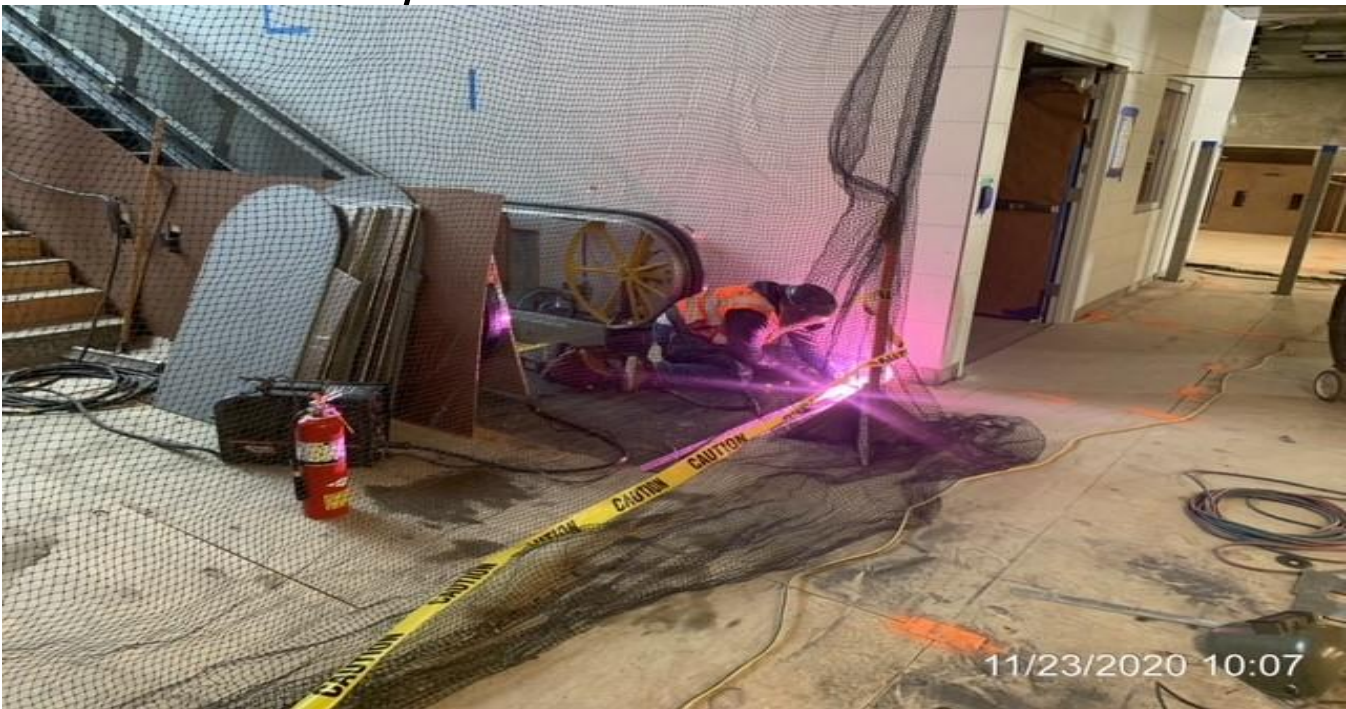
MLK STATION – Continue installing steel mud pans to the edges of Escalators 1&2 at the concourse.
