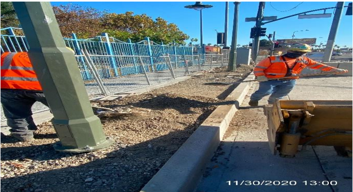
LEIMERT PARK STATION – Fine grading sidewalk on northbound Crenshaw Blvd between Vernon Ave and 43rd Pl.
