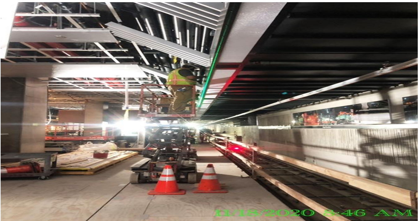
EXPO STATION – Installing down stand support plate to the edge lights along the southbound of the platform.
