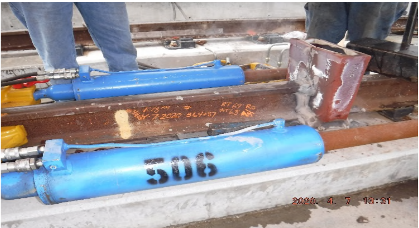
48 th Street - STA 364+87 TK#3-SB looking west – right rail de-stress weld (48th St)
