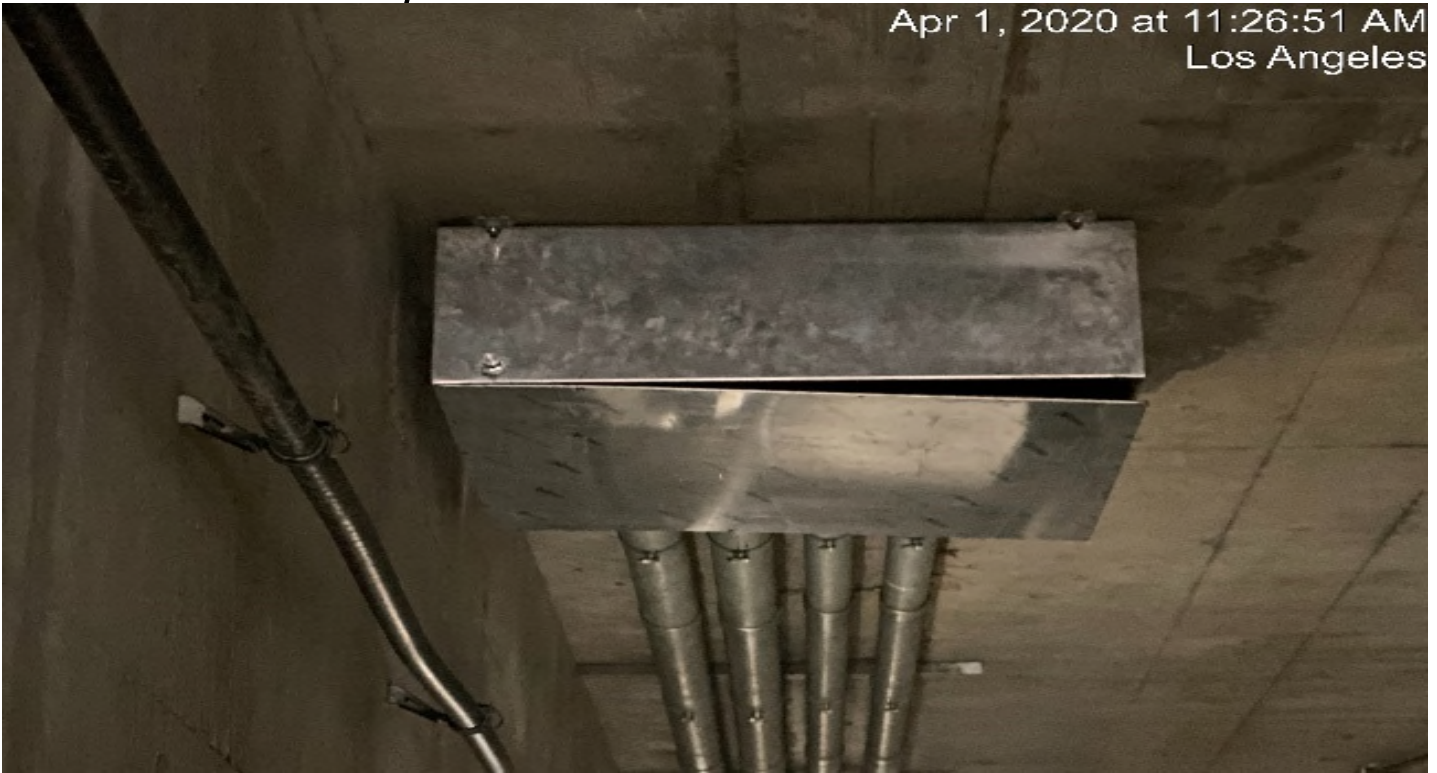
UG3 – DCD adjusting pull box southbound UG-3.
