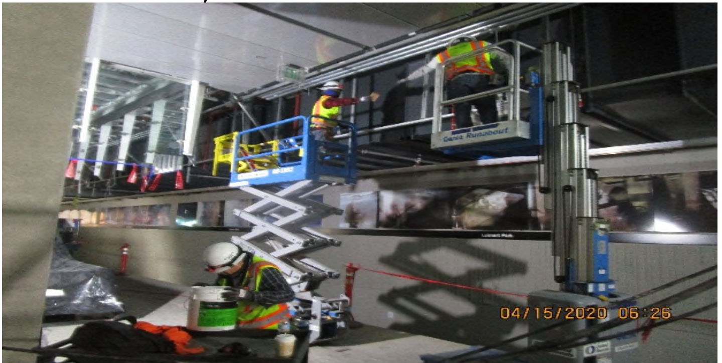
Crenshaw/Vernon - South platform, northbound continued rough in Radiax cable 2" GRC conduit & support racks.
