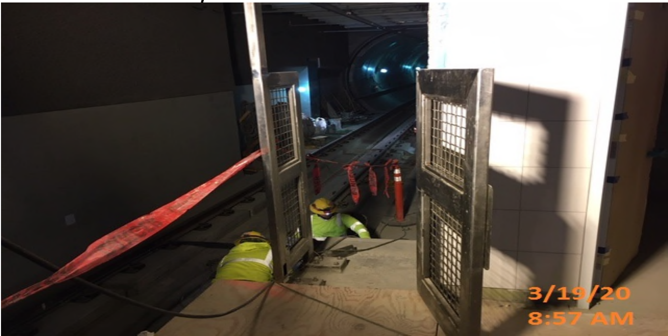
LEIMERT PARK STATION – Installing end gates for the southbound stair landing on the north end of the platform level.
