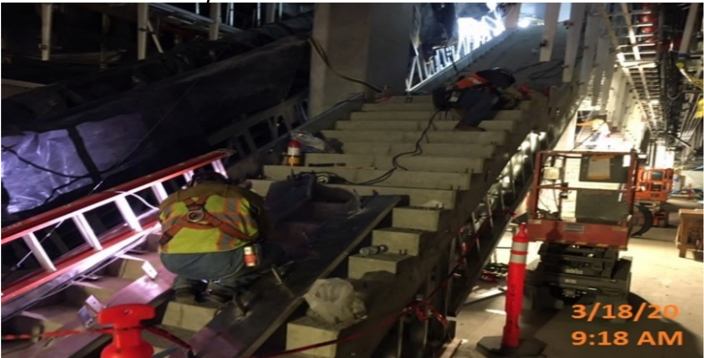
MLK STATION – Installing anchor tabs for the edge plate installation for stairwell #2 between concourse and platform level.
