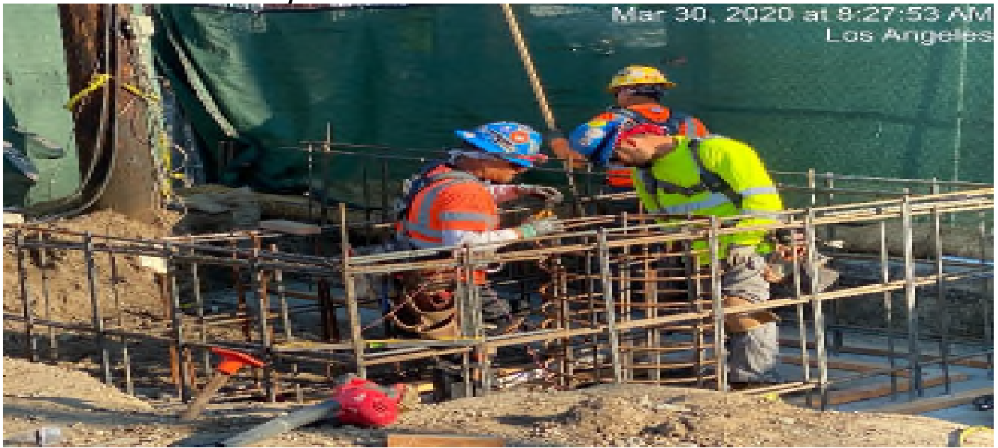
LEIMERT PARK STATION – Continue rebar installation for the planar wall and footings at the east side of the plaza level.
