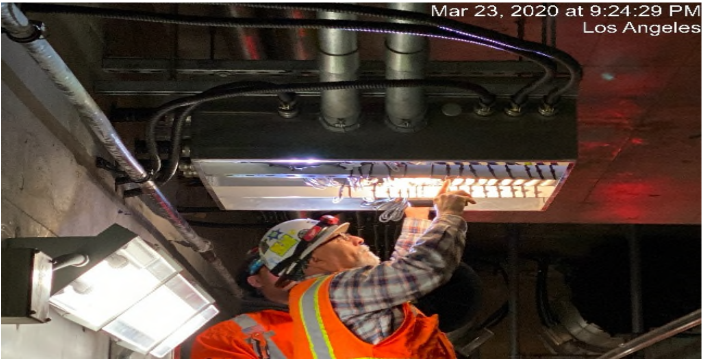
UG3 – Continue grounding wires for the tunnel booster junction boxes at the southbound tunnel at Sta 291+50.
