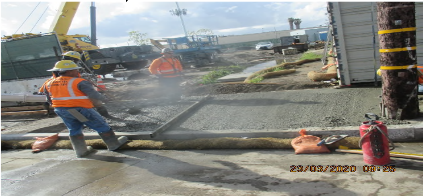
UG3 – Placing concrete for the new sidewalk/driveway installation on the southwest corner of 67th St and Crenshaw Blvd. 3/23/20
