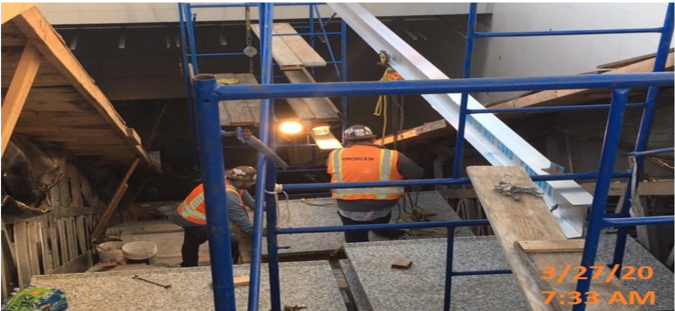
MLK STATION – Continue moving granite landing sections into place for installation at the main entrance structure of the plaza level.
