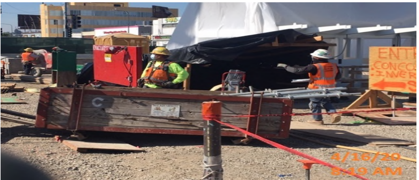
EXPO STATION – Setting up materials to build scaffold and platform for Elevator shafts 1&2 at the plaza level.
