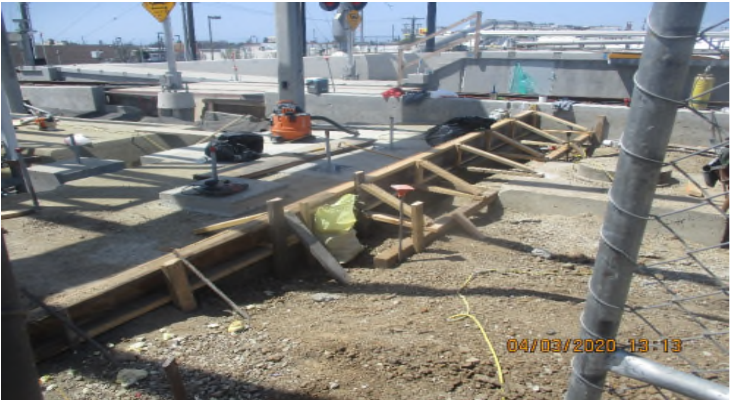
Florence/Brea – WSCC Carpenters formed for plaza platform at s-ticket pavilion La Brea Station.
