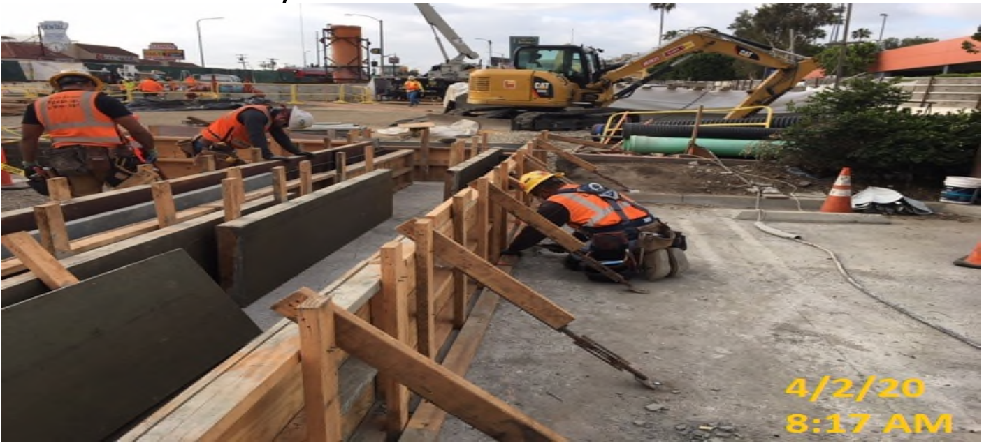
MLK STATION – Continue formwork for the planter wall installation at the west side of the plaza level.
