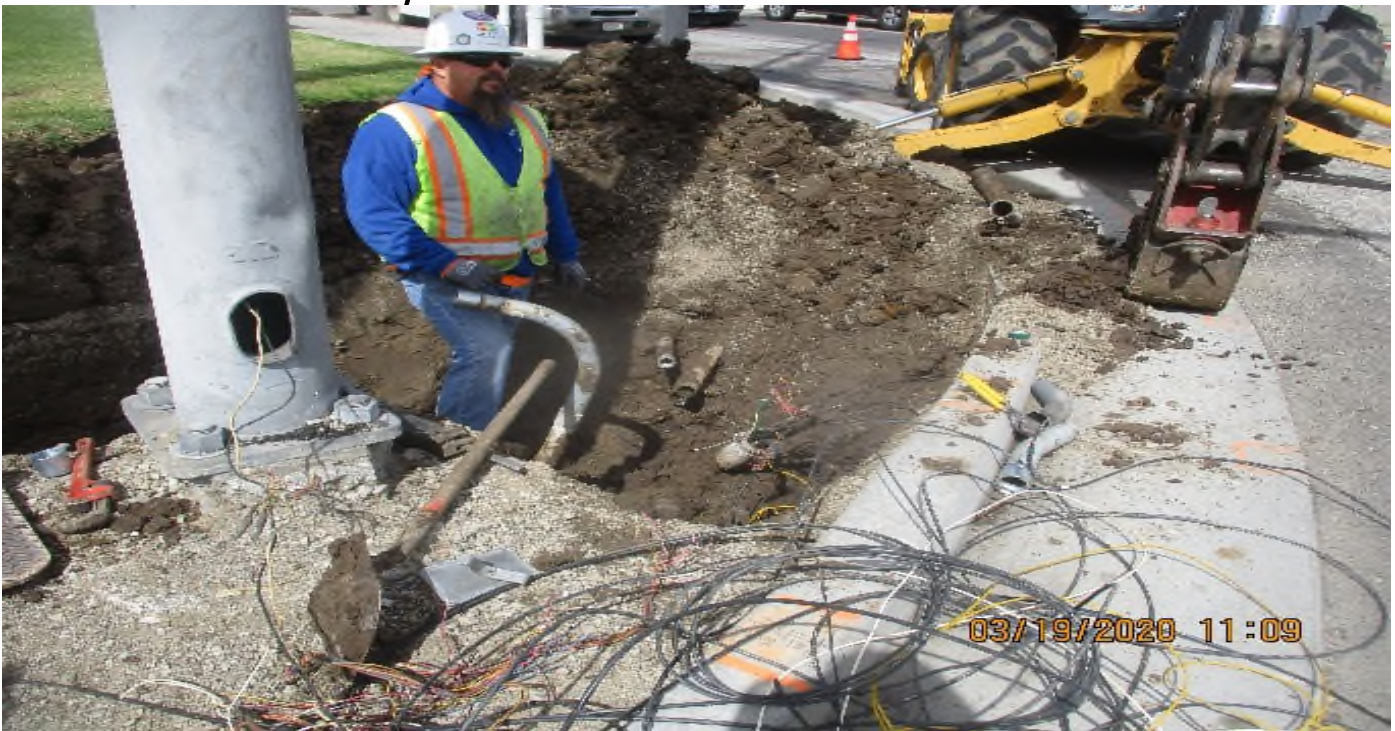
Aviation/Century – Select Electric Relocating pull boxes away from ADA ramp at S/W cor of Manchester and Aviation.
