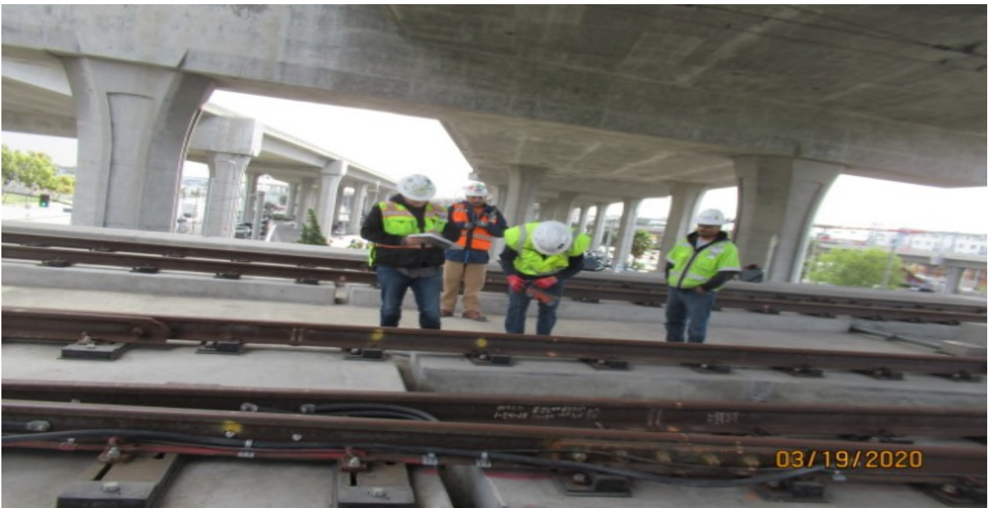
WSSC & RMA- Site Scan, ex-ray of ends of plinths at GL Wye (looking east)
