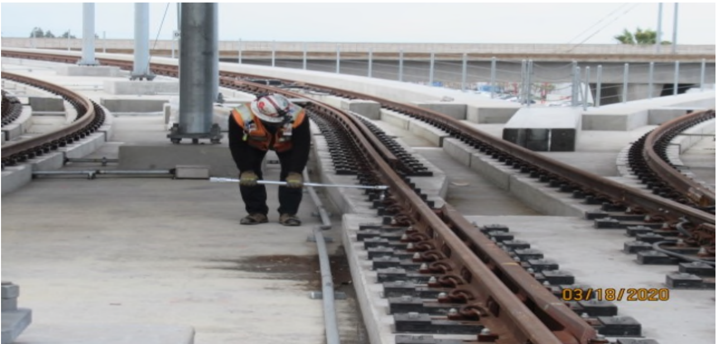
WSSC QC track inspector, verifying 300 FT. lbs. of torque on DF fastener bolts on PTSB 2300 at GL Wye STA 12+95
