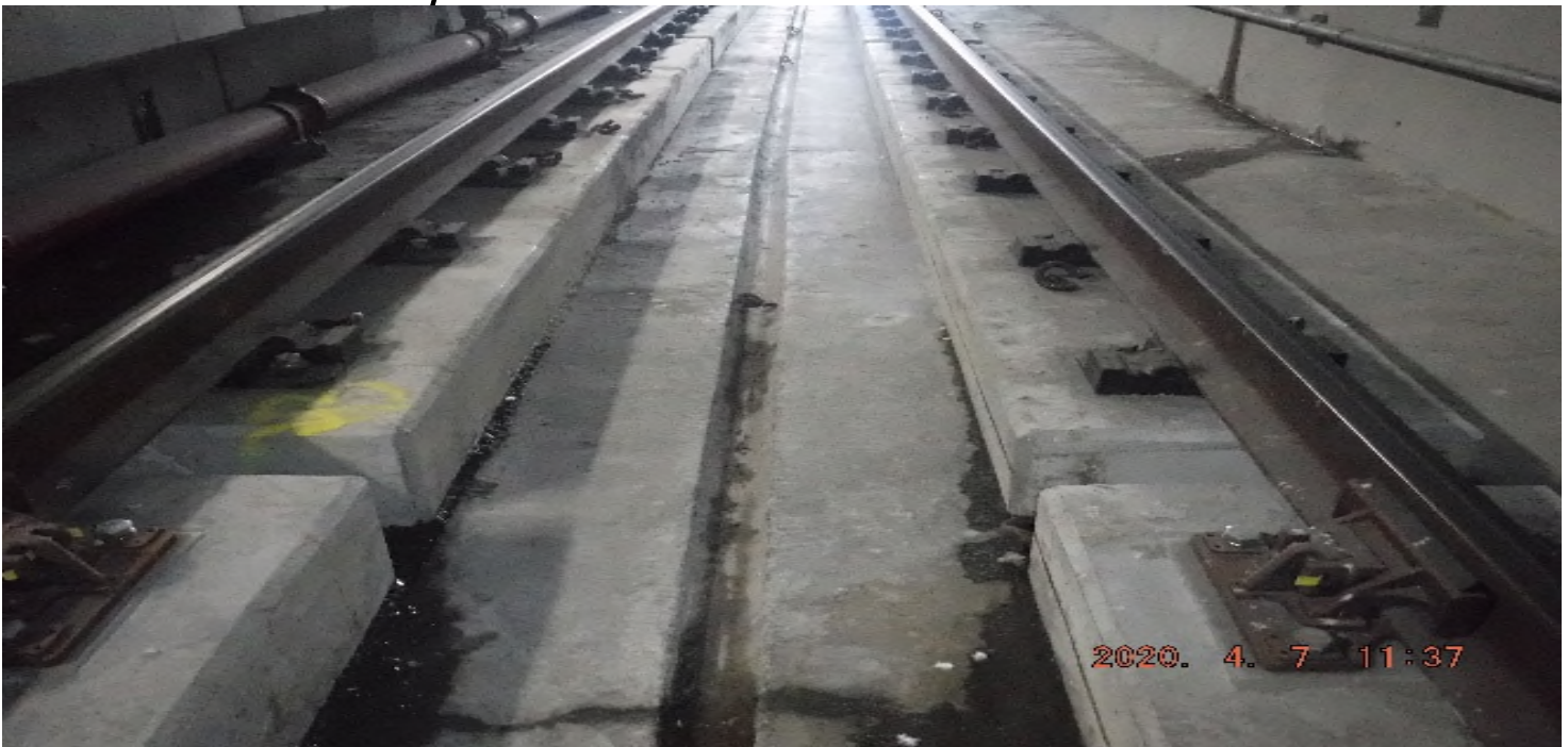
UG4 – STA 372+50 TK#3-SB looking south – north lim of rail de-stress @ VHRF (UG4 48th St-Vernon)
