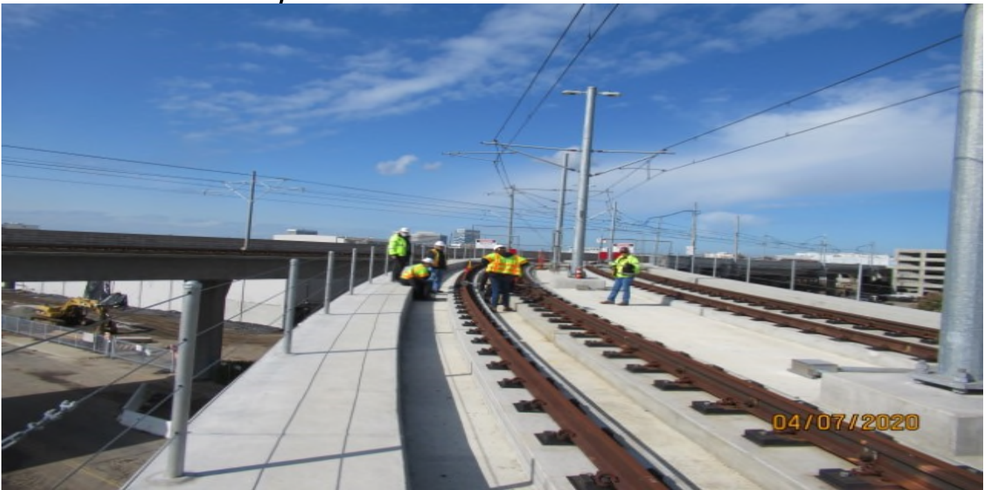
Guideway - GL Wye NBW 2310 STA 10+36 Metro-WSCC site walk for rail profile radius verification.
