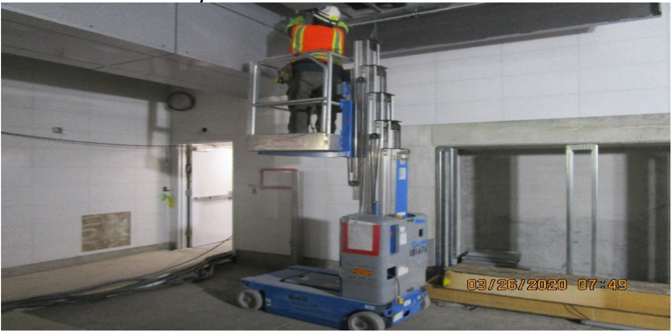
MLK STATION – Continue installing light cove and ceiling panels throughout the Free & Paid Area of the concourse level.
