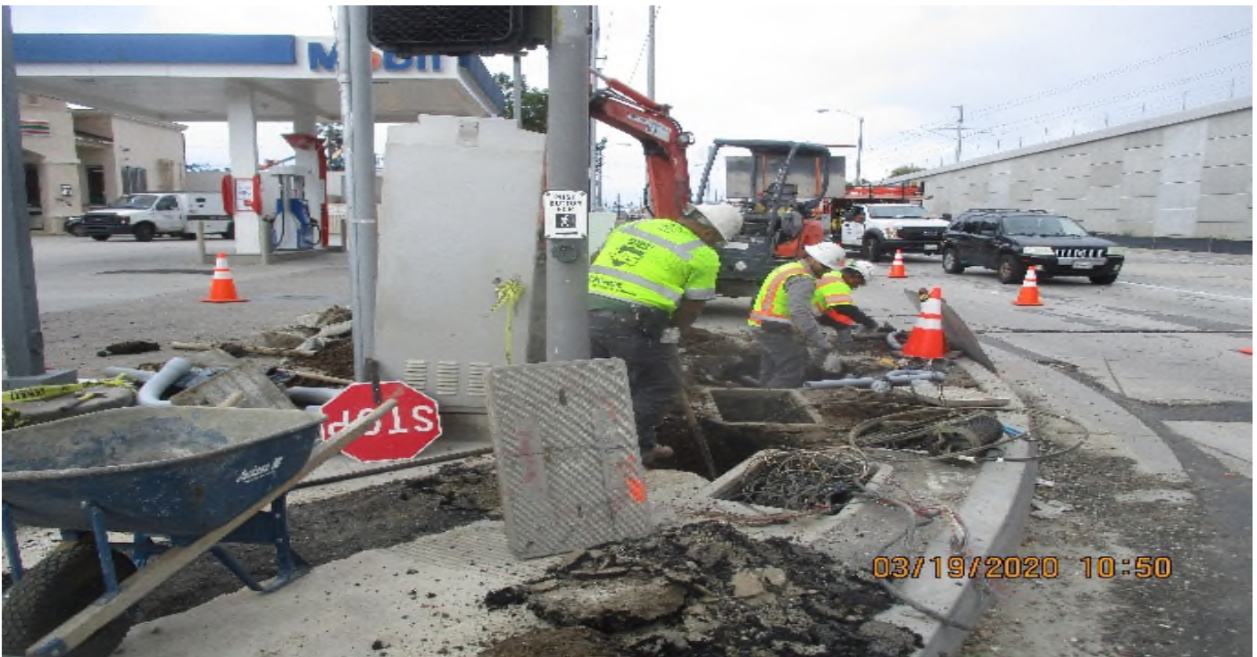
Aviation/Century – VT Electric Excavating trench for TS conduit at Manchester and Aviation.
