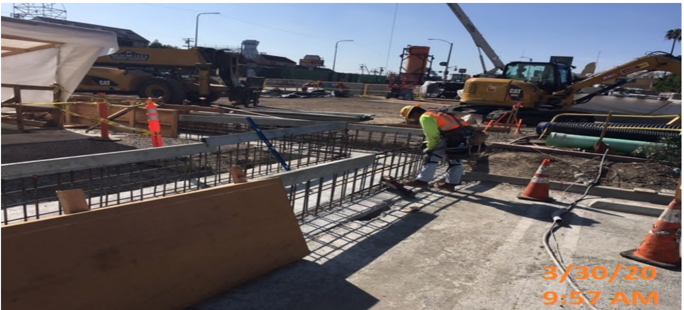
MLK STATION – Continue planter wall and footing installation at the west side of the plaza level.
