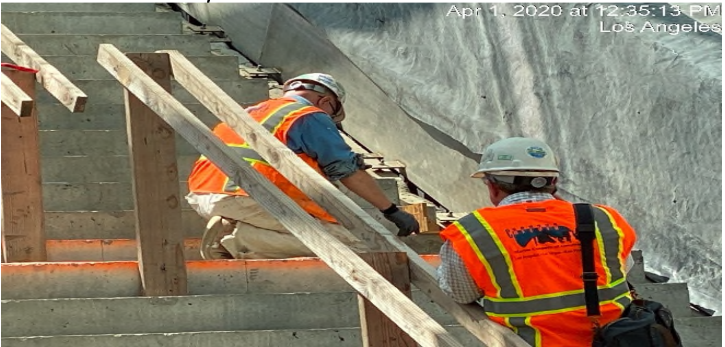
LEIMERT PARK STATION – Began layout for granite installation at the main stair case landing of the plaza level.
