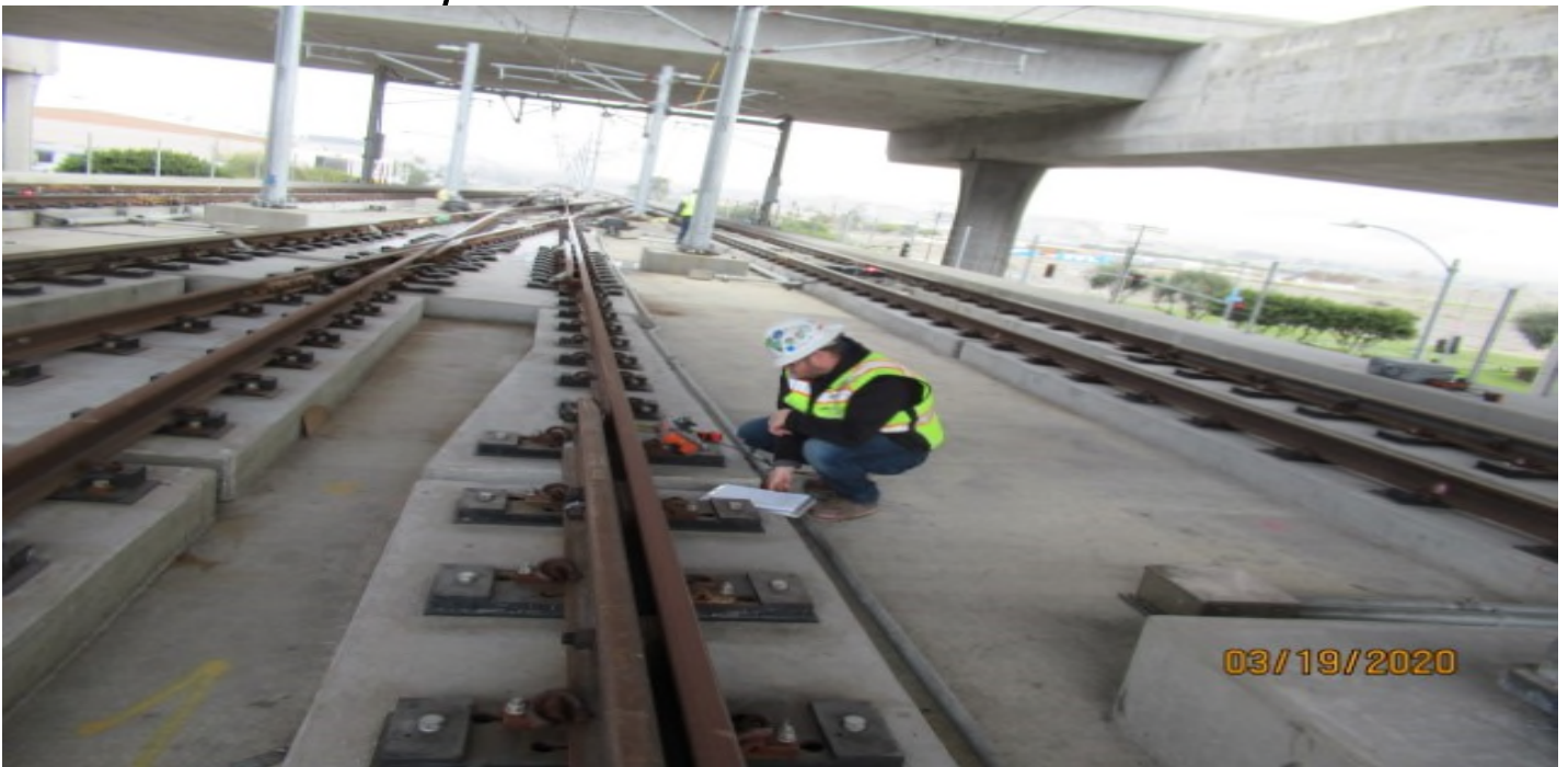
RMA-Site Scan inspector on SB2300 PT STA 12+92 GL Wye, ex-ray of rebar dowel location to invert (looking north)
