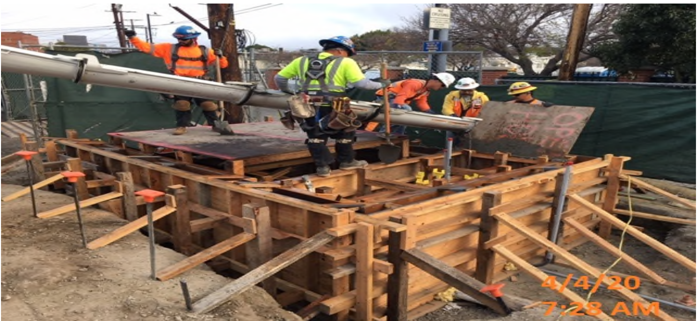
LEIMERT PARK STATION – Placing concrete for the planar wall at the east side of the plaza level.
