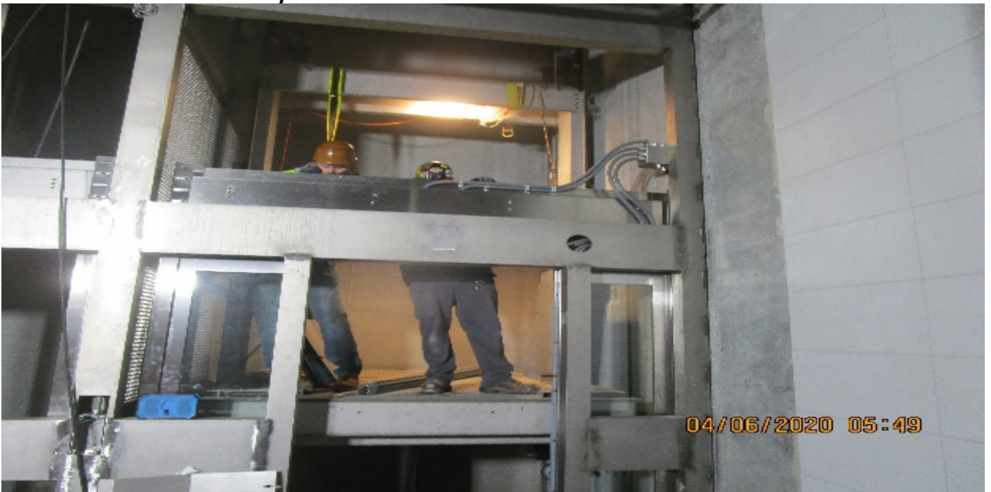
Crenshaw/MLK - MLK Concourse, Elevator 1 & 2 Cabs, Continued rough in stainless steel finish facia panels.
