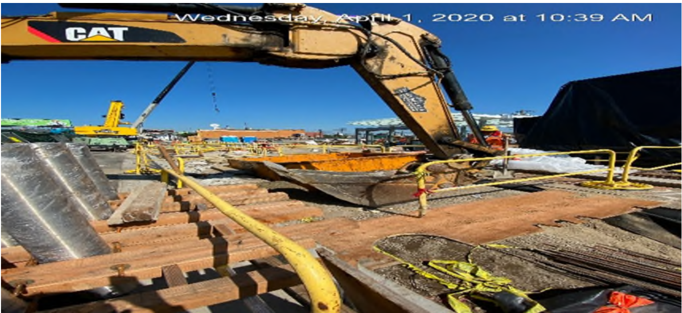
LEIMERT PARK STATION – Excavating for DWP water line adjacent to the southeast corner of Crenshaw Blvd and 43rd Pl.
