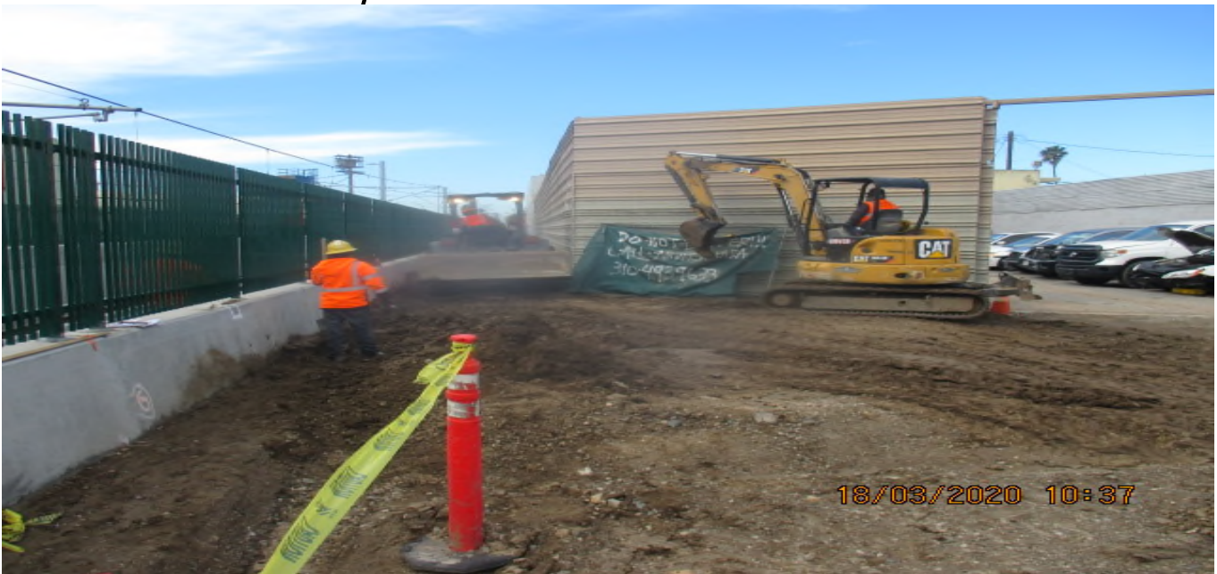
UG3 – Continued excavating/grading for the culvert drainage installation along the southbound barrier wall in preparation for concrete placement. 3/18/20
