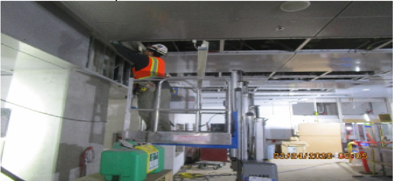
MLK STATION – Continue installing light cove and ceiling panels throughout the Free & Paid Area of the concourse level.
