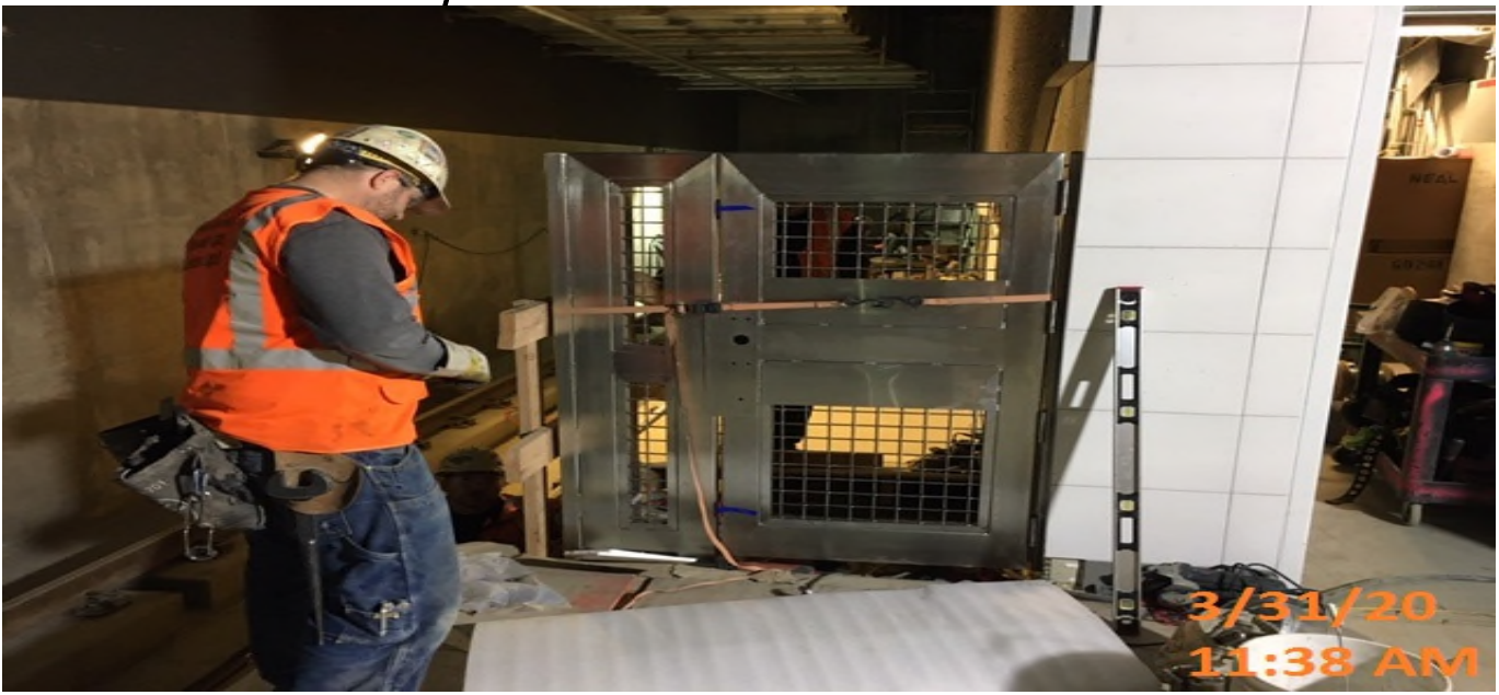
LEIMERT PARK STATION – Installing end gates for the southbound stair landing on the north end of the platform level.
