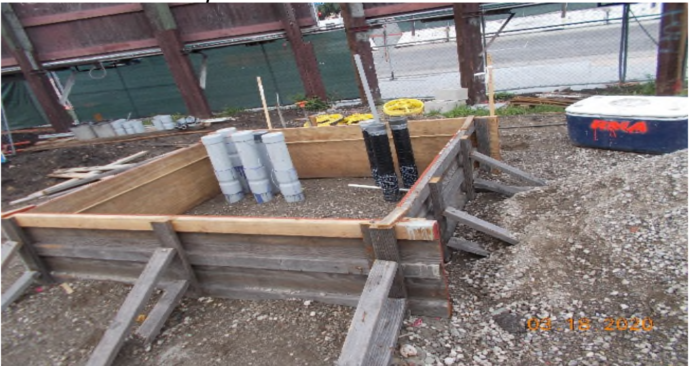
PARK MESA – Raising DWP meter sections in preparation for concrete placement of meter pad at TPSS#7 on 60th St & Crenshaw Blvd.
