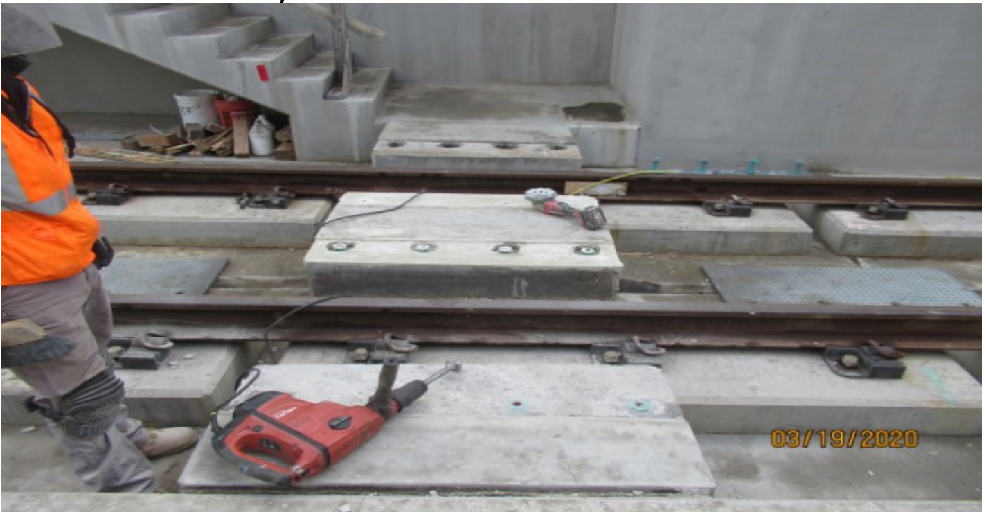
UG – 1 - WSCC Bushing & grinding out concrete foundations for Ped. Crossings on NB #4 track in UG1 STA 56+50 (looking east)
