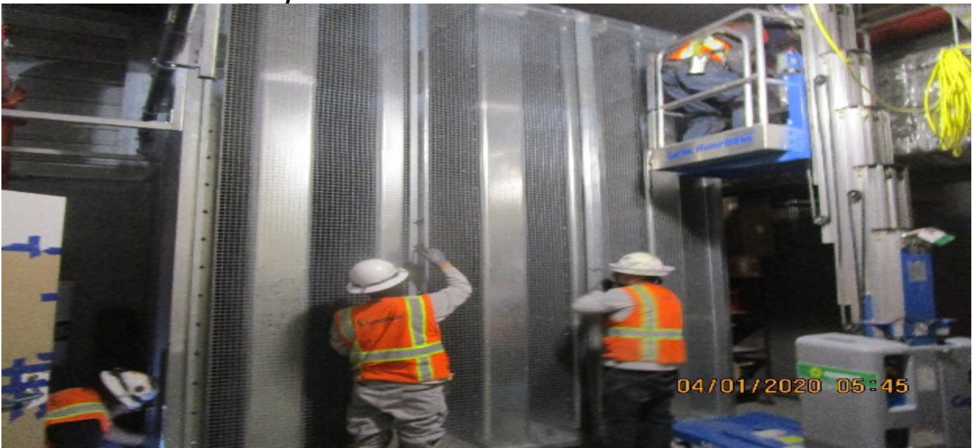
LEIMERT PARK STATION – Installing bird screen protection for the sound attenuator for EVF-6-301 in the South Fan Room C – 102 of the concourse level.
