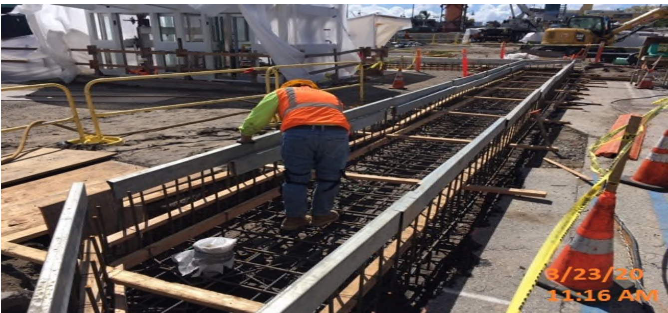
MLK STATION – Continue planter wall and footing installation at the west side of the plaza level.
