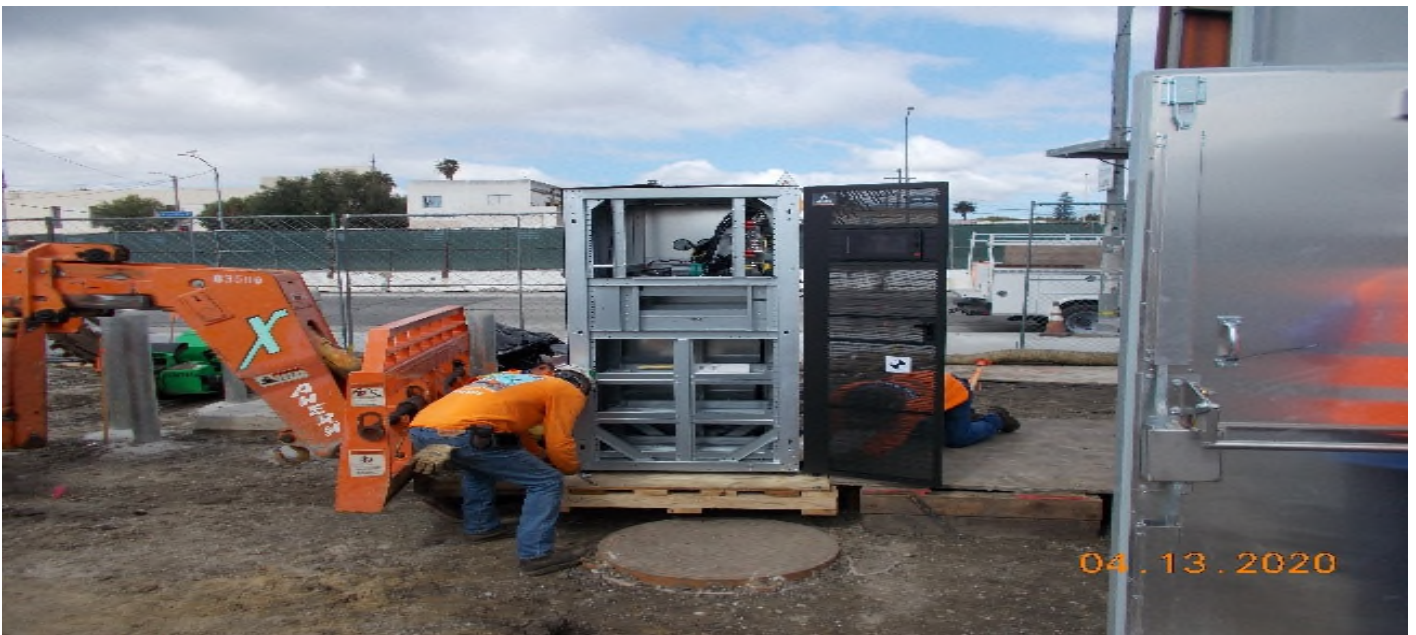
PARK MESA – Began installing UPS equipment inside the Auxiliary Power Bungalow at TPSS#7 on 60th St & Crenshaw Blvd.
