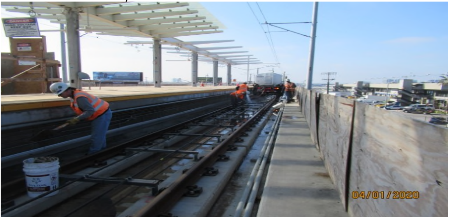
Aviation/Century – HCC on Century-Aviation bridge SB #3 track, cleaning bridge deck (looking south)
