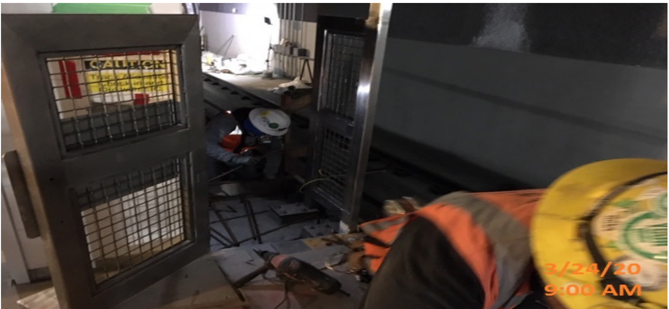
LEIMERT PARK STATION – Continue end gate installation for the southbound stair landing on the south end of the platform level.
