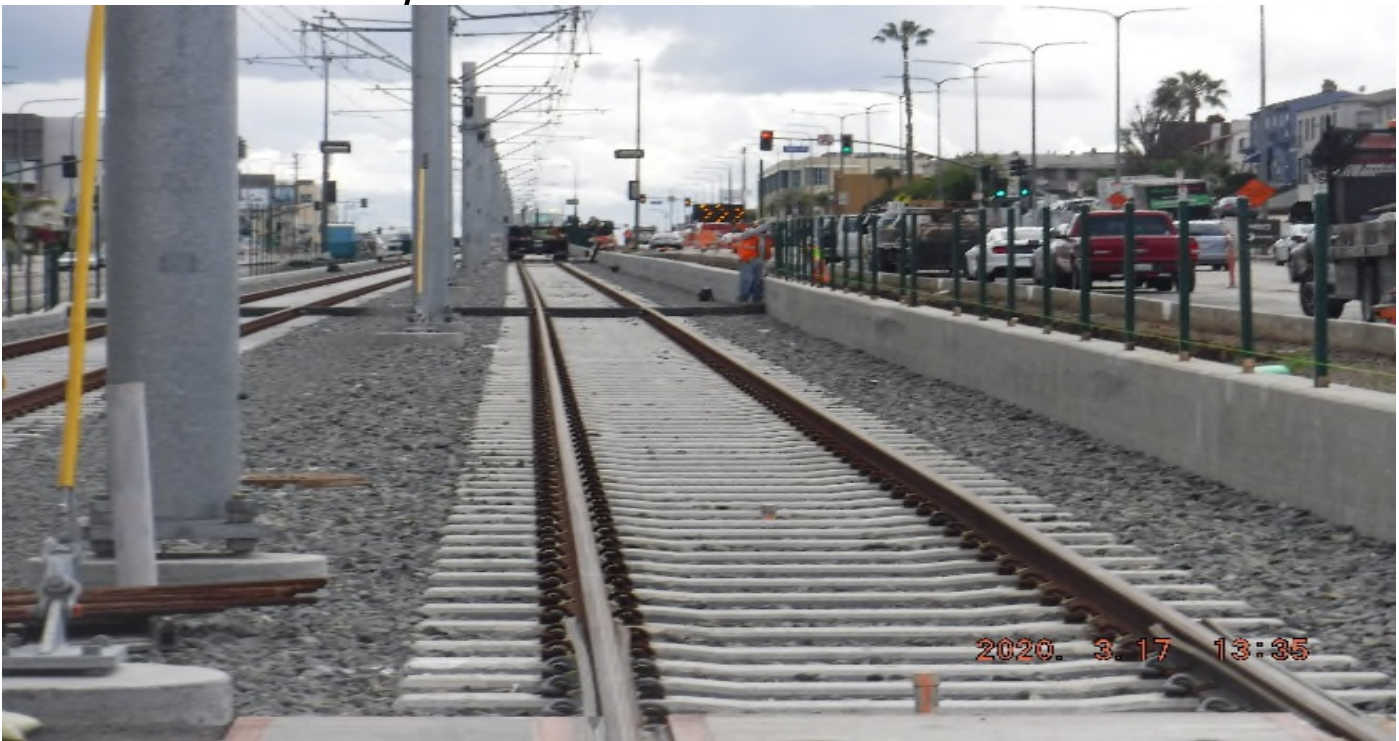
48 th Street - STA 363+00 TK#3. SB looking south – fence work SB ballast wall, south of 48th St.
