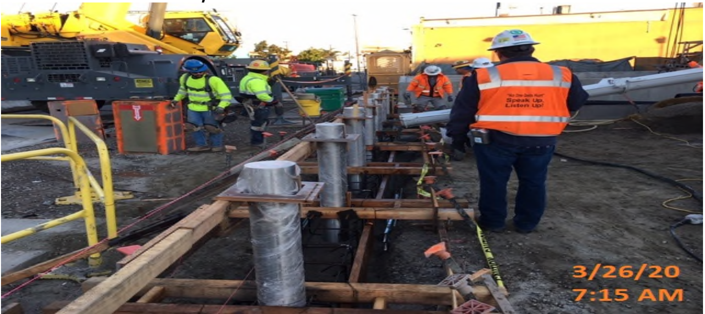
LEIMERT PARK STATION – Placing concrete for the stainless steel station bollards at the west edge of the plaza level.
