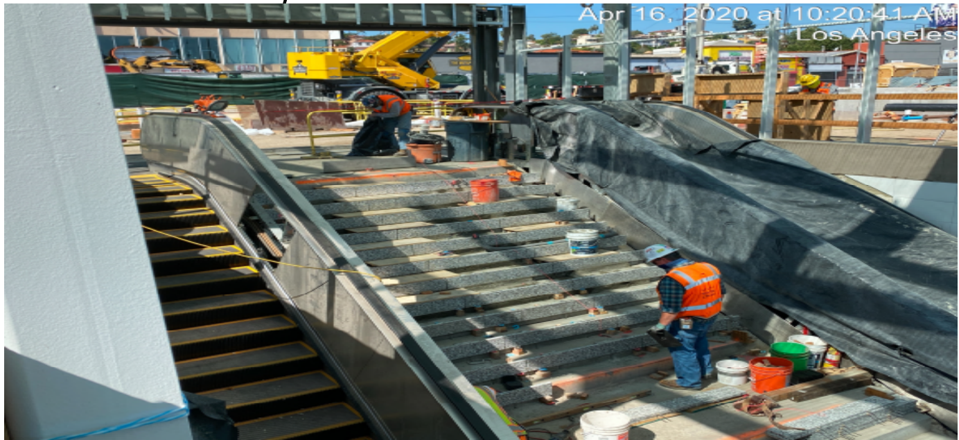
LEIMERT PARK STATION – Continue granite thread and riser installation at the main stair case landing of the plaza level.
