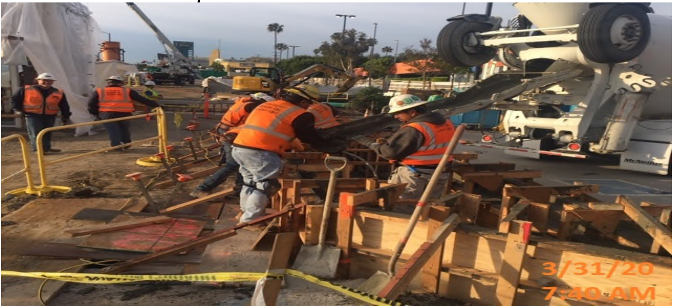
MLK STATION – Placing concrete for the planter wall and footing installation at the west side of the plaza level.
