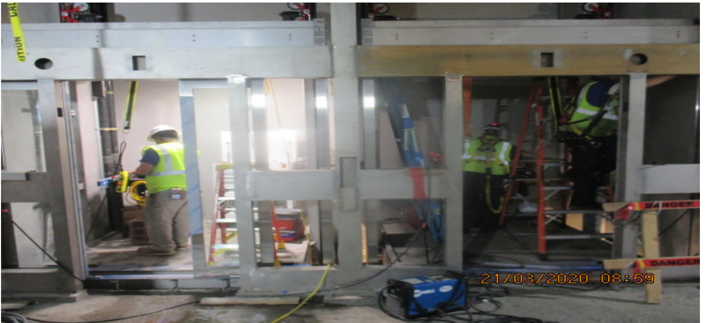
MLK STATION – Began installing door mechanisms for Elevators 1 – 4 at the concourse level.
