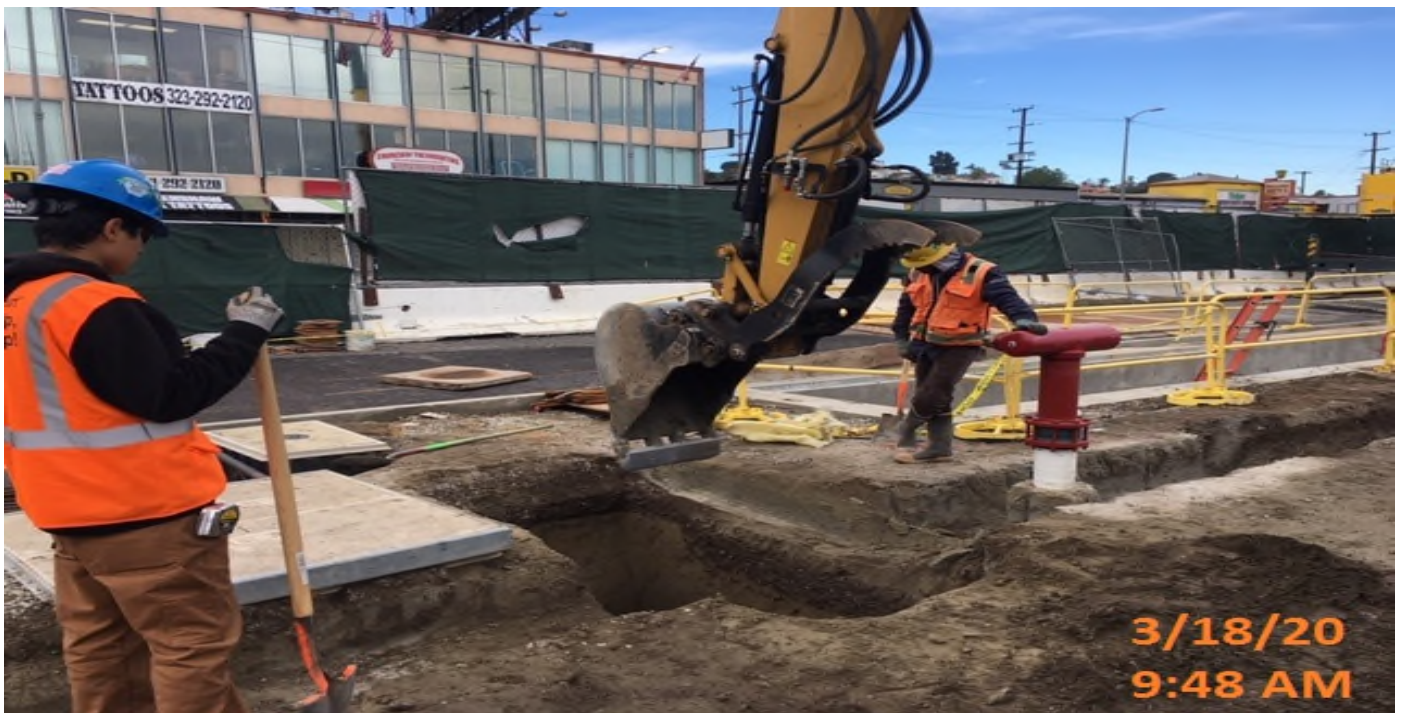
Crenshaw/Vernon - WSCC crew exploratory excavating for water leak into station mechanical room.
