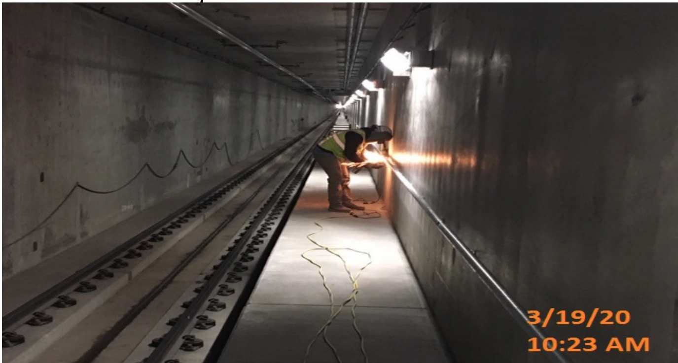
UG3 – Continue installing and welding handrails for the emergency walkway at the southbound tunnel from Sta 288+45 – 290+60.
