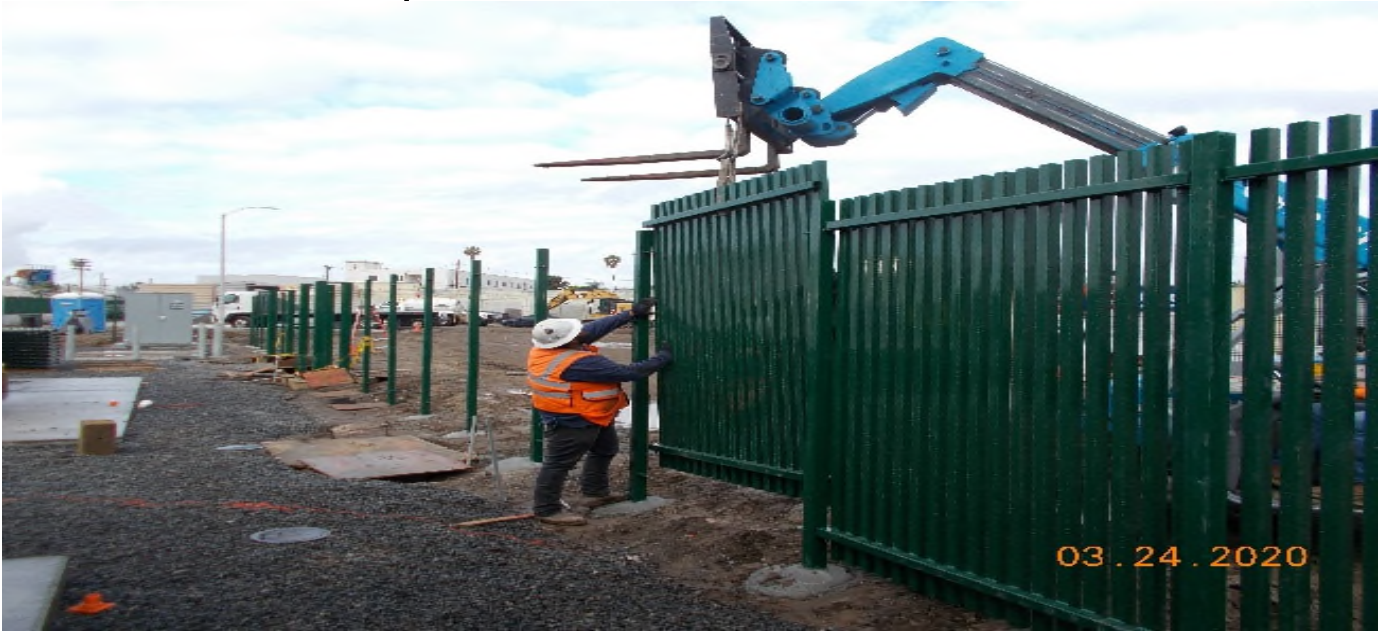
UG3 – Continue installing fence posts around the Auxiliary power site perimeter adjacent to the south end portal entrance.
