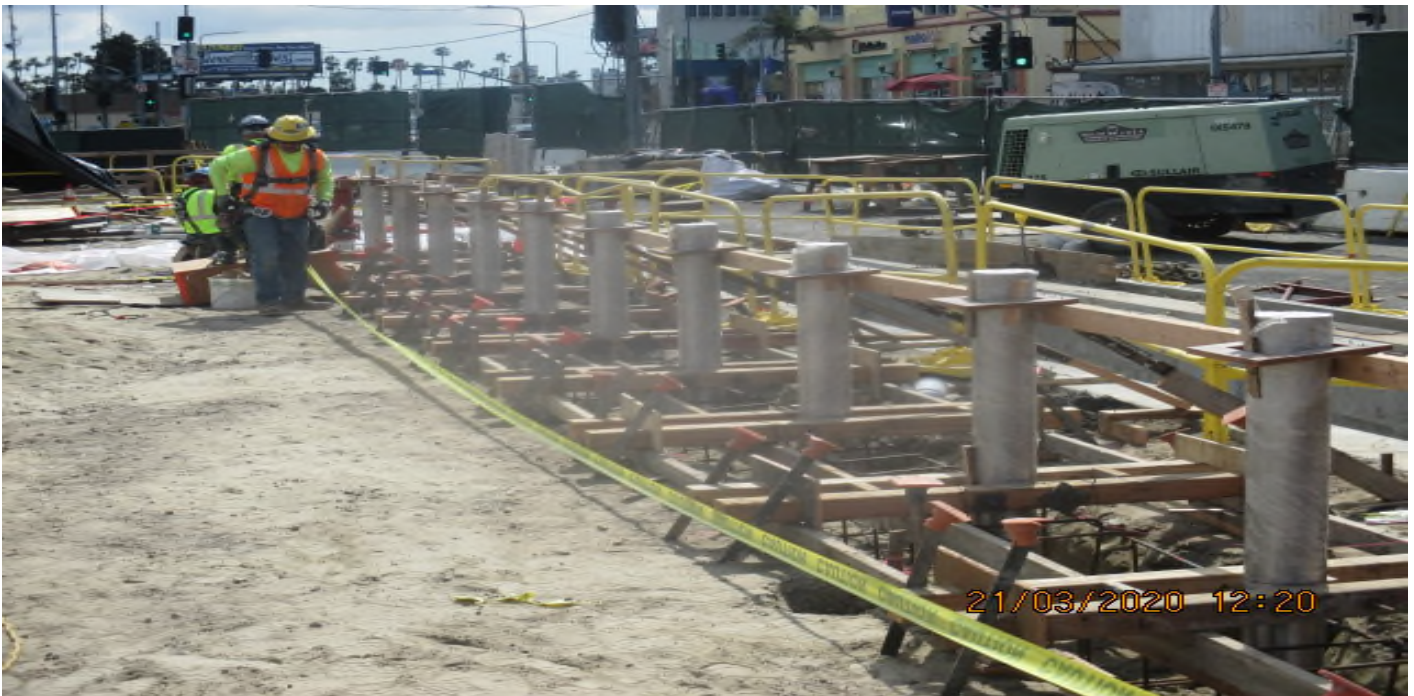
LEIMERT PARK STATION – Installing stainless steel station bollards at the west edge of the plaza level. 3/21/20
