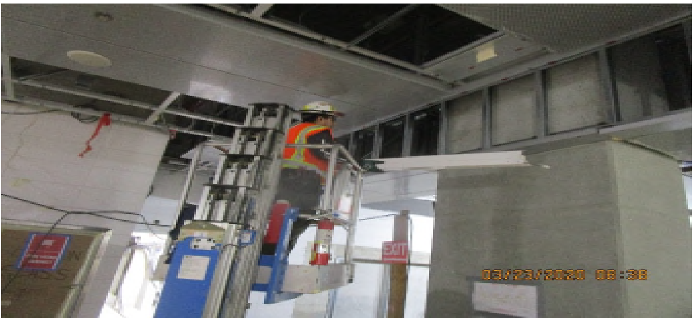
MLK STATION – Continue installing light cove and ceiling panels throughout the Free & Paid Area of the concourse level.
