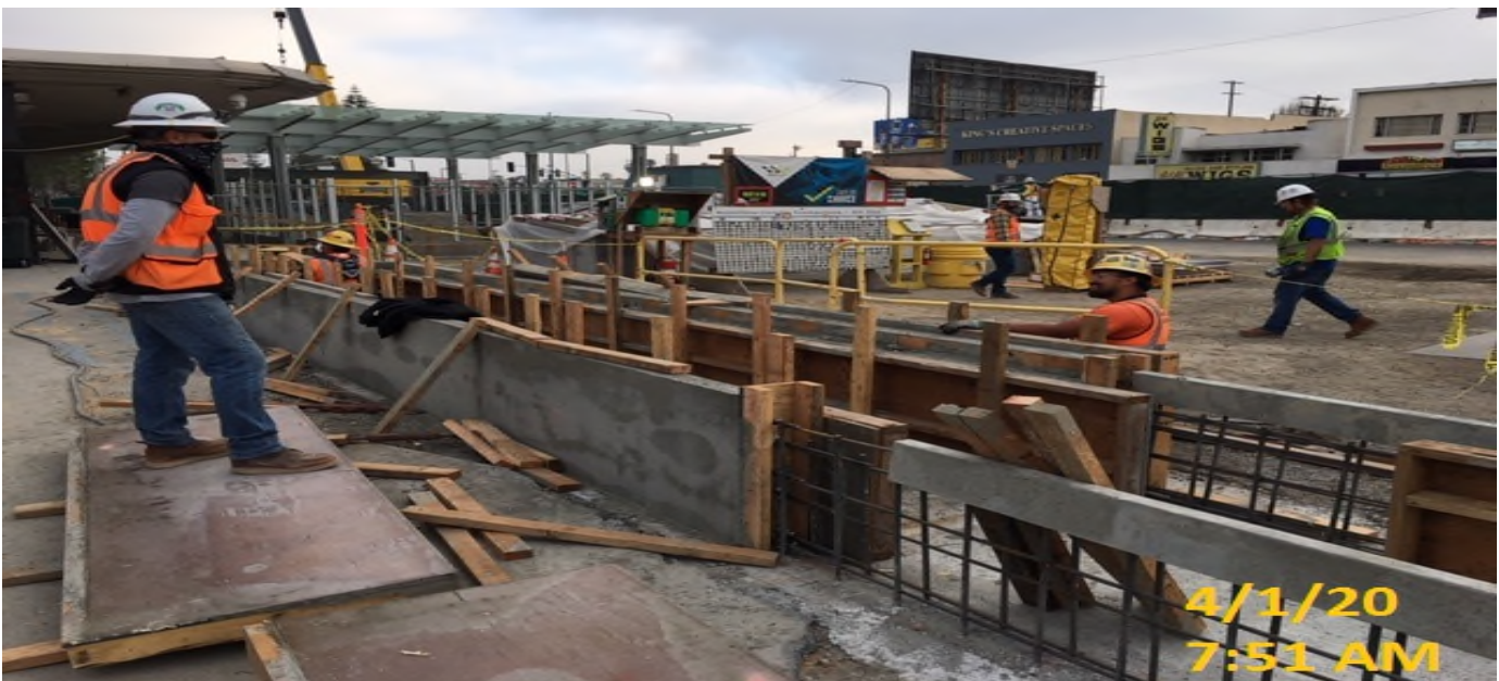
MLK STATION – Continue formwork for the planter wall installation at the west side of the plaza level.
