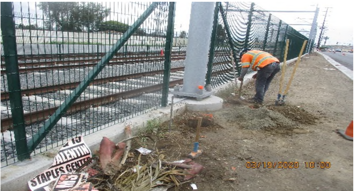
Florence/High St. - ACE Fence Dig holes for posts at East Bound Florence W-High.
