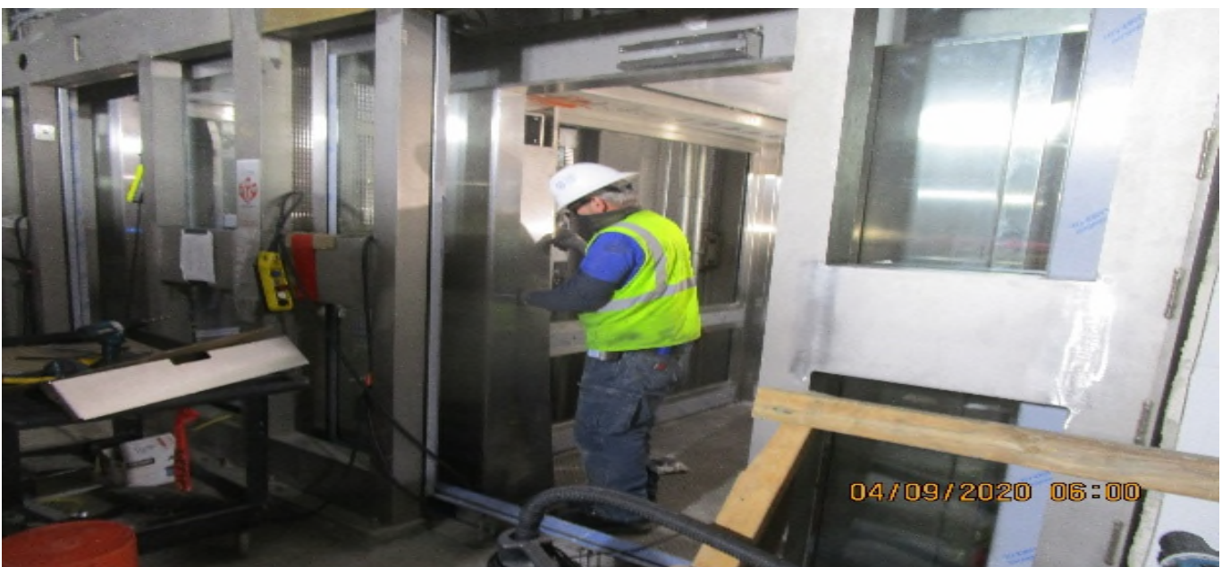
MLK STATION – Continue cab assembly and stainless steel fascia panel installation for all the Elevators at the concourse level.
