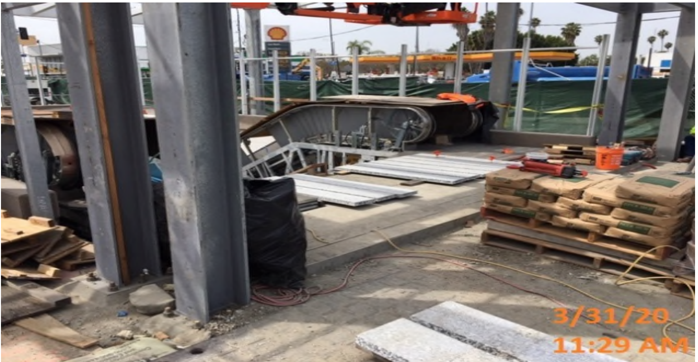
EXPO STATION – Continue installing granite stair treads at the main entrance staircase landing of the plaza level.
