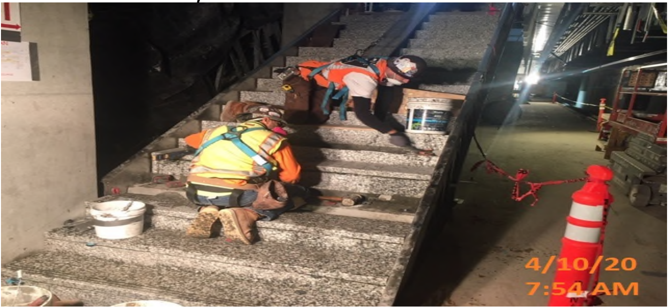
MLK STATION – Continue installing granite risers for staircase #3 between concourse and platform level.
