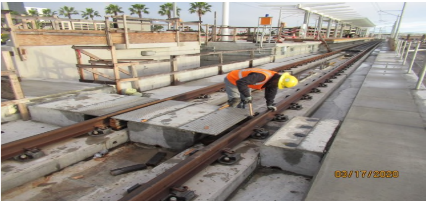
Aviation/Century – WSCC labor removing galvanized plate from Ped. Crossing on NB #4 track on Century.Aviation Bridge STA 66+18 Rework
