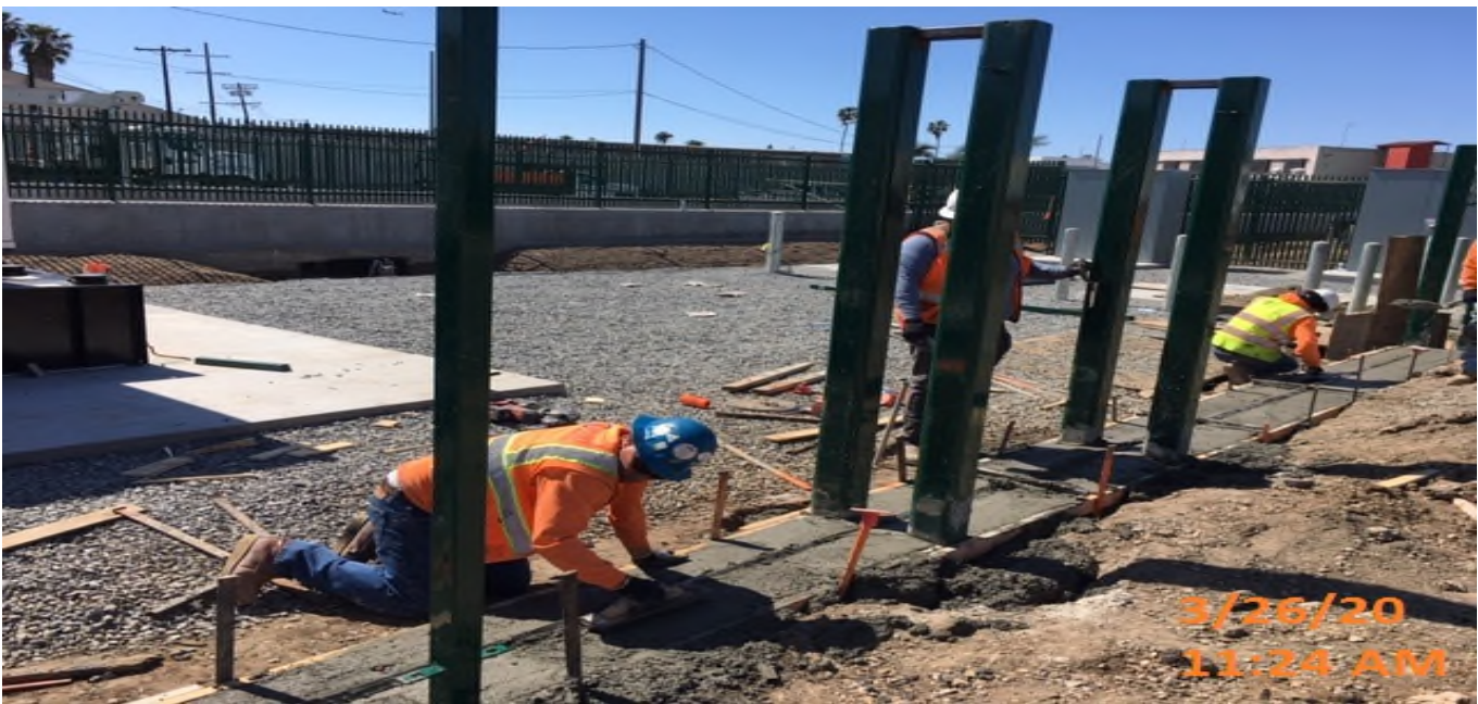
UG3 – Continue installing fence posts and floor channel for sliding fence gate around the Auxiliary power site perimeter adjacent to the south end portal entrance.
