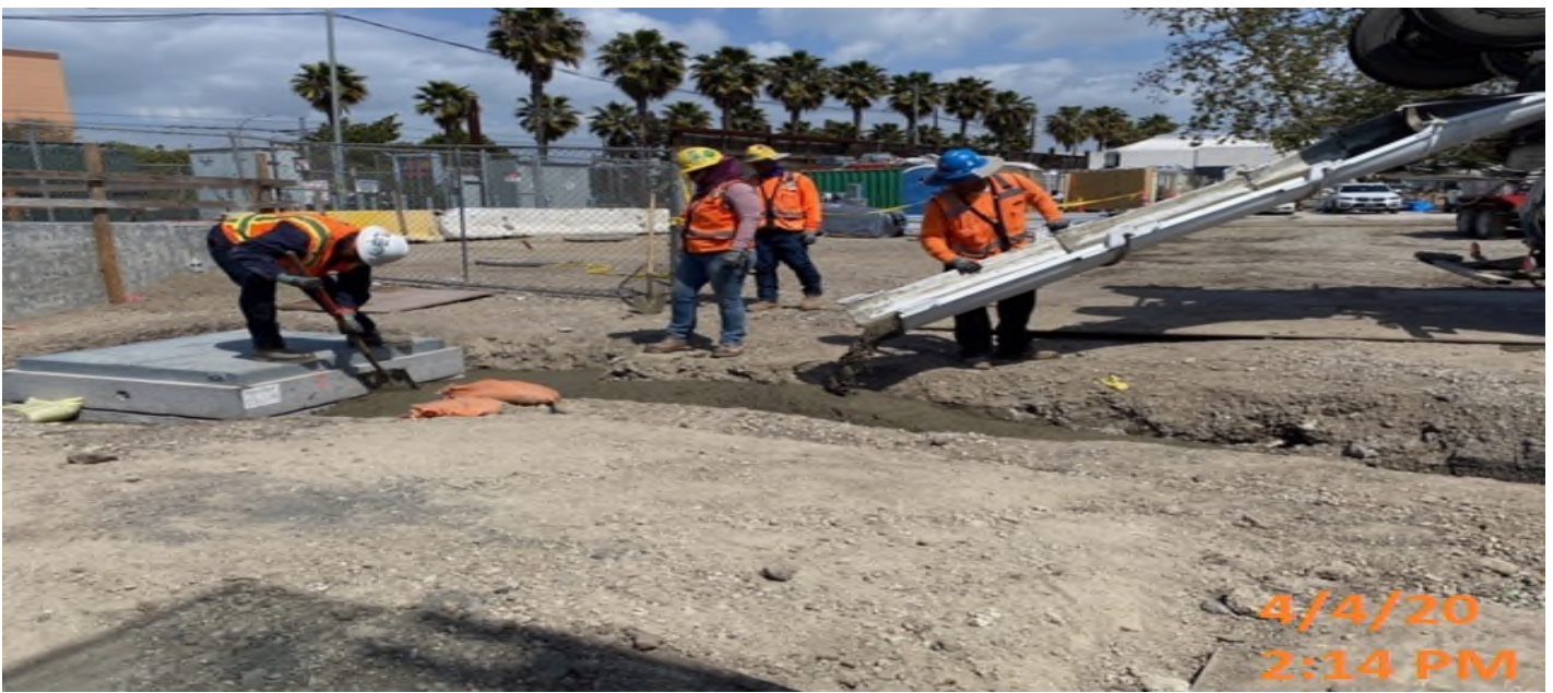
EXPO STATION – Continue fiber-tie in installation and placing slurry for the electrical duct banks M02 & M07 at the plaza level.
