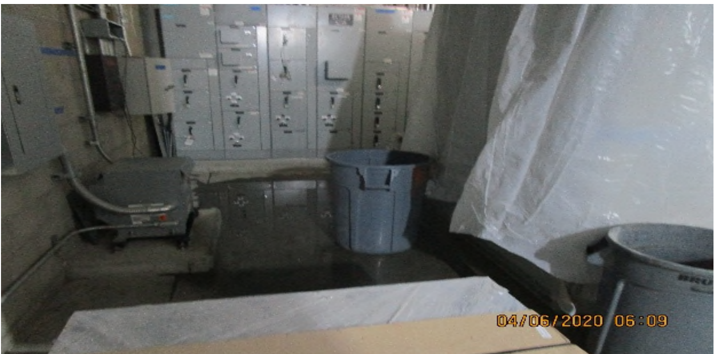
Crenshaw/MLK - MLK, Aux Power (N) C132, southside PX1-N, Overhead water intrusion from embedded 12"x12" comm JB-34.
