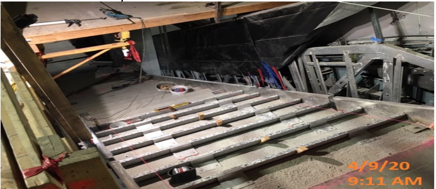
EXPO STATION – Began installing granite risers for staircase #2 at the concourse level.
