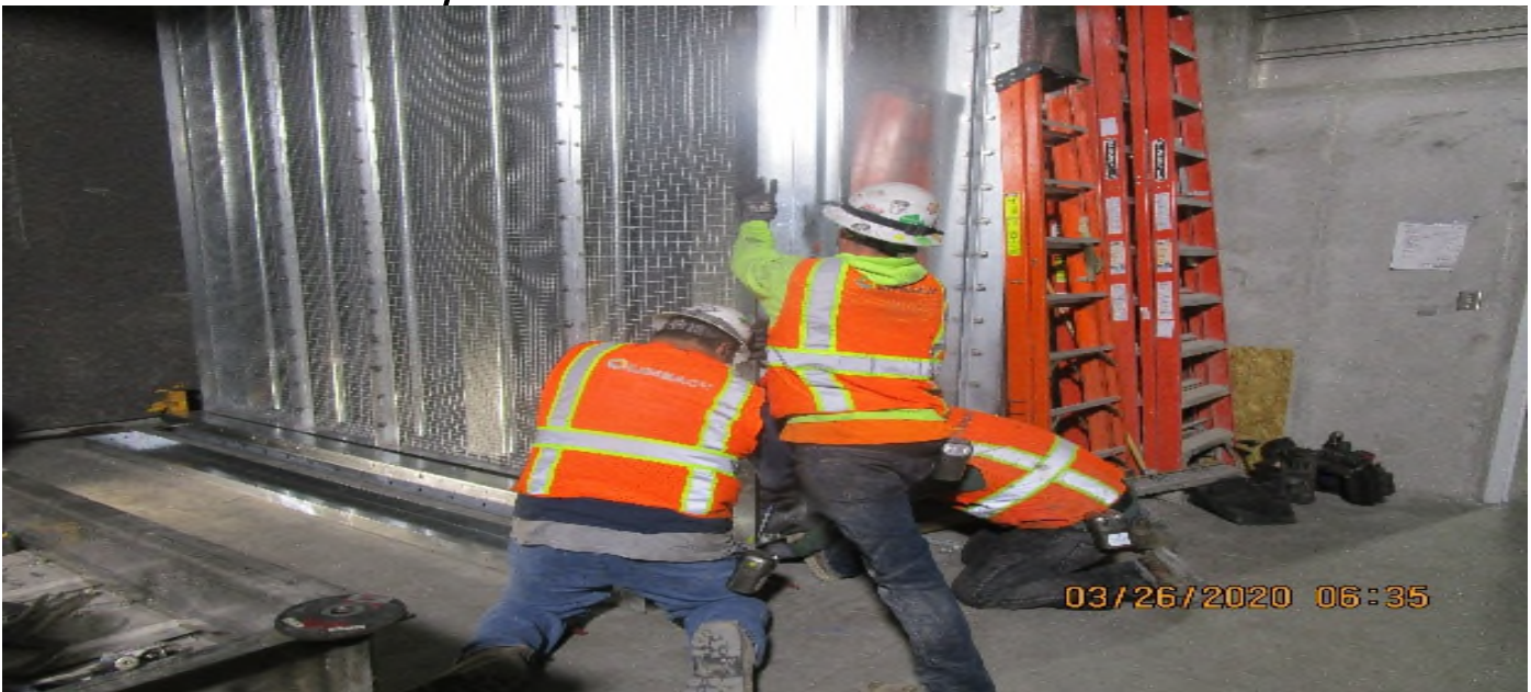
LEIMERT PARK STATION – Continue tunnel fan damper section installation for the sound attenuator for EVF-6-102 in the North Fan Room C – 142 of the concourse level.
