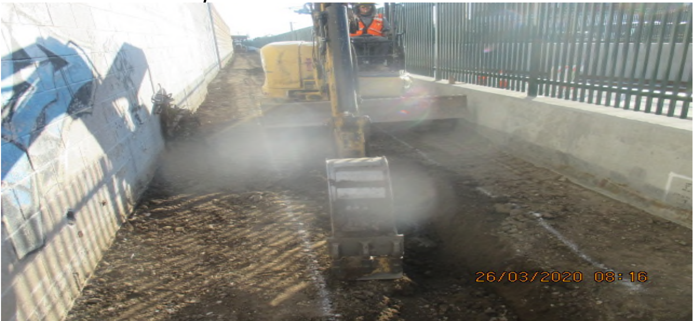
UG3 – Continue excavating for culvert drainage along the bottom of the southbound barrier wall in preparation for concrete placement. 3/26/20
