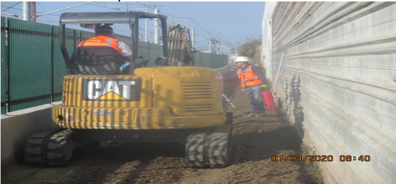
UG3 – Continue excavating for culvert drainage along the bottom of the southbound barrier wall in preparation for concrete placement. 4/1/20
