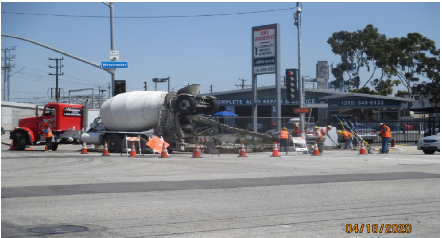
Manchester Bridge – Placing concrete for the ADA ramp at Manchester and Florence.
