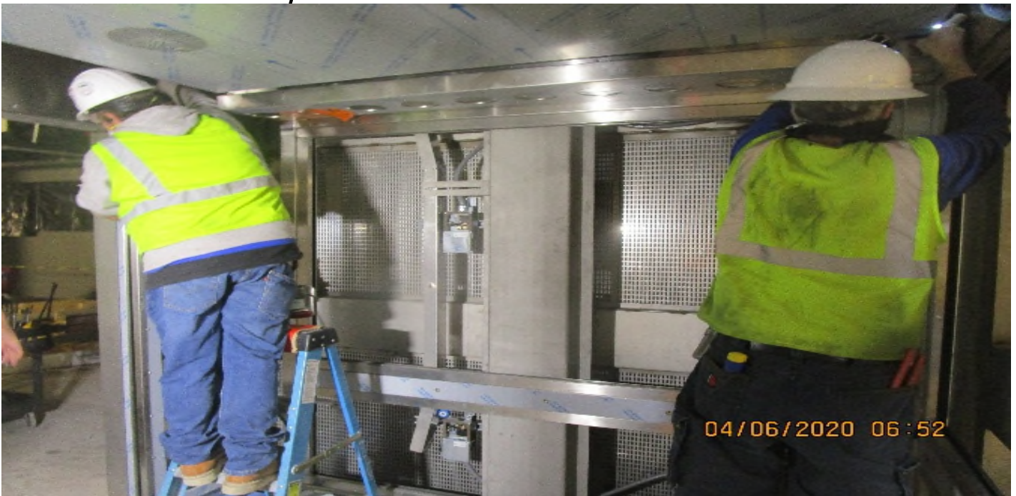
MLK STATION – Continue cab assembly and stainless steel fascia panel installation for Elevators 3&4 at the concourse level.
