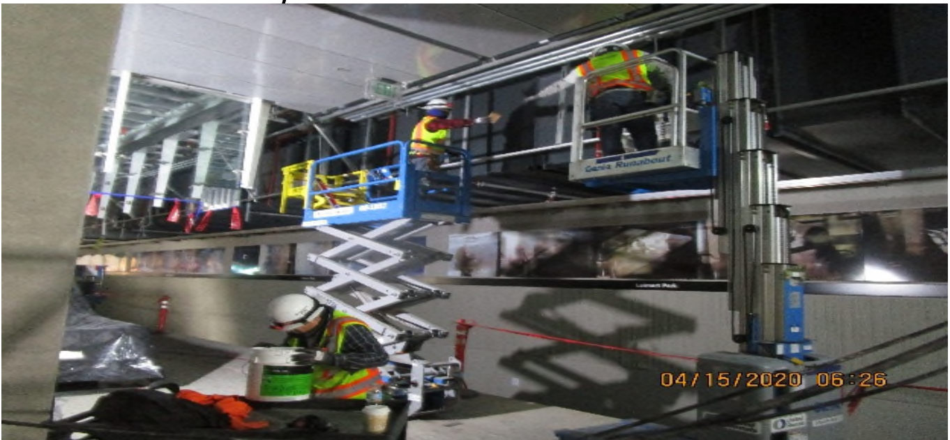
LEIMERT PARK STATION – Continue radiax cable conduit and support rack installation on the platform ceiling level.
