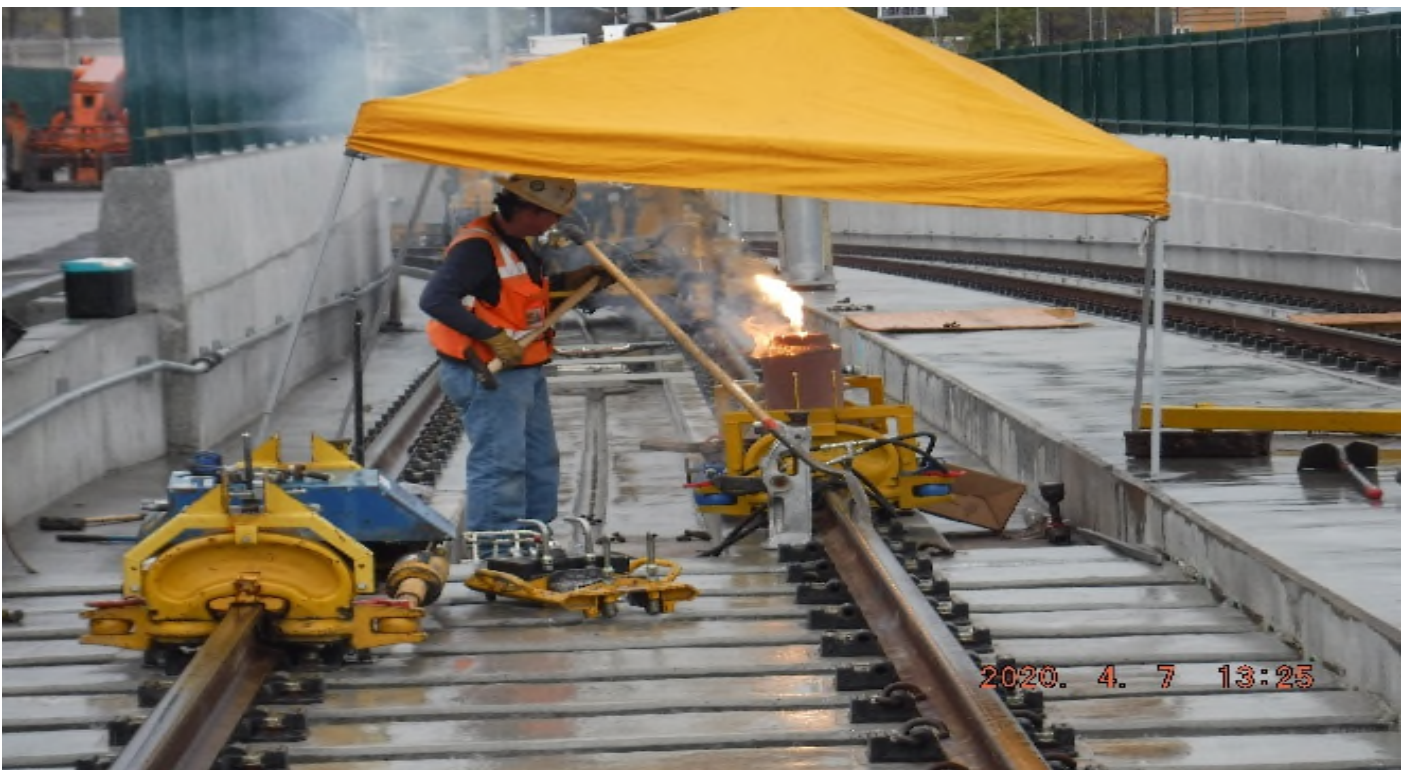
48 th Street - STA 364+87 TK#3-SB looking north – right rail de-stress weld in progress.
