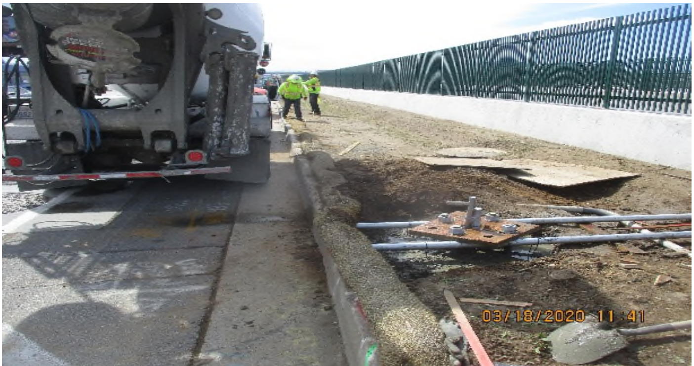
111 th Street – DB Electric Placing Concrete SL and TS foundations at 111th and 104th street.
