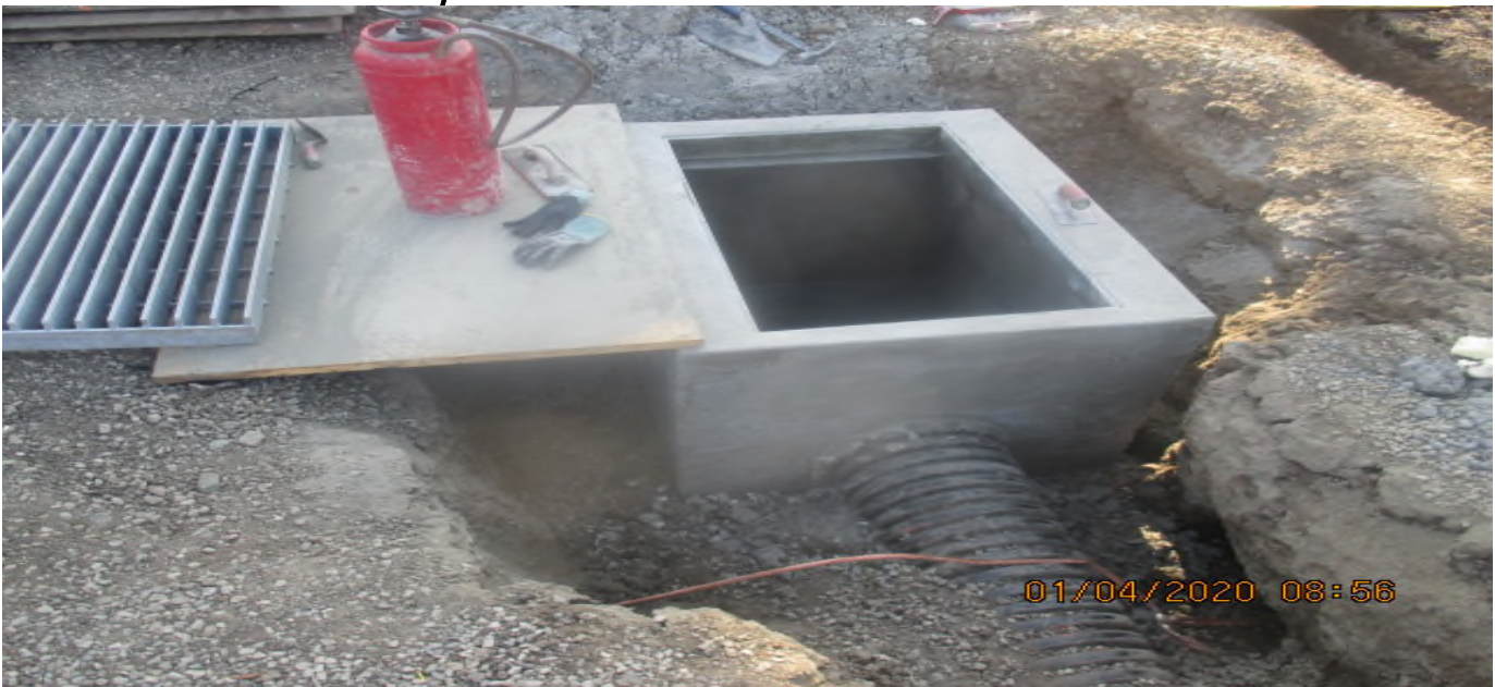
PARK MESA – Sack and patching inlet structure N-12 at TPSS#7 on 60th St & Crenshaw Blvd. 4/1/20
