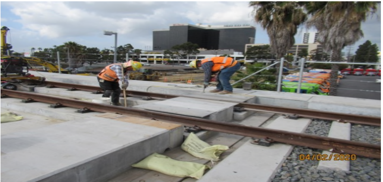
Aviation/Century – WSCC working on emergency walkway foundations Century-Aviation bridge SB #3 track STA 74+60 (looking west) Rework
