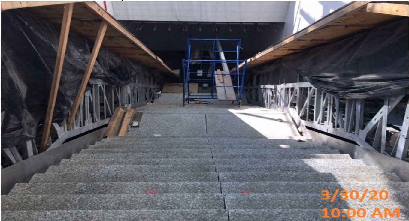
MLK STATION – Completed granite installation at the main entrance structure of the plaza level.
