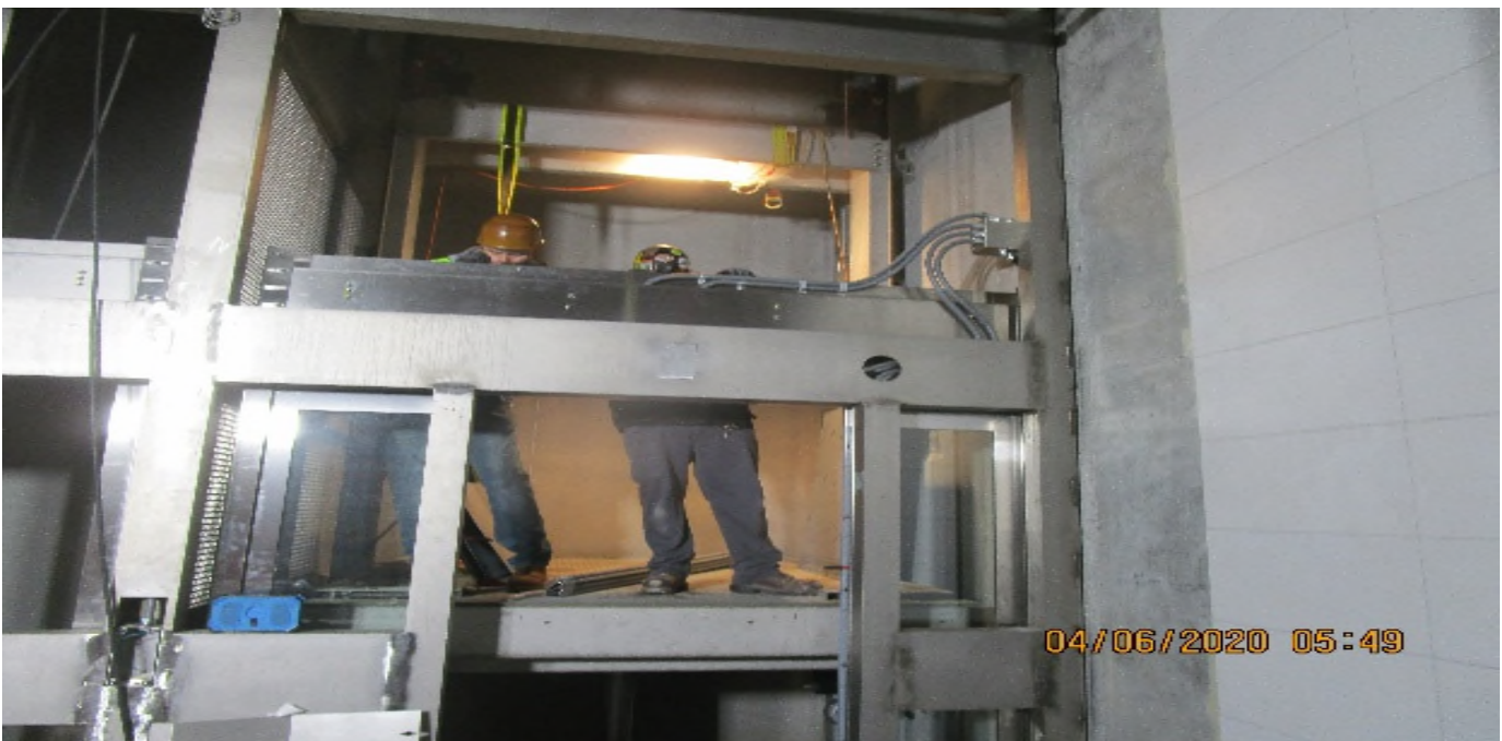
MLK STATION – Continue cab assembly and stainless steel fascia panel installation for Elevators 1&2 at the concourse level.
