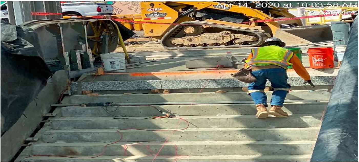
LEIMERT PARK STATION – Continue granite thread and riser installation at the main stair case landing of the plaza level.
