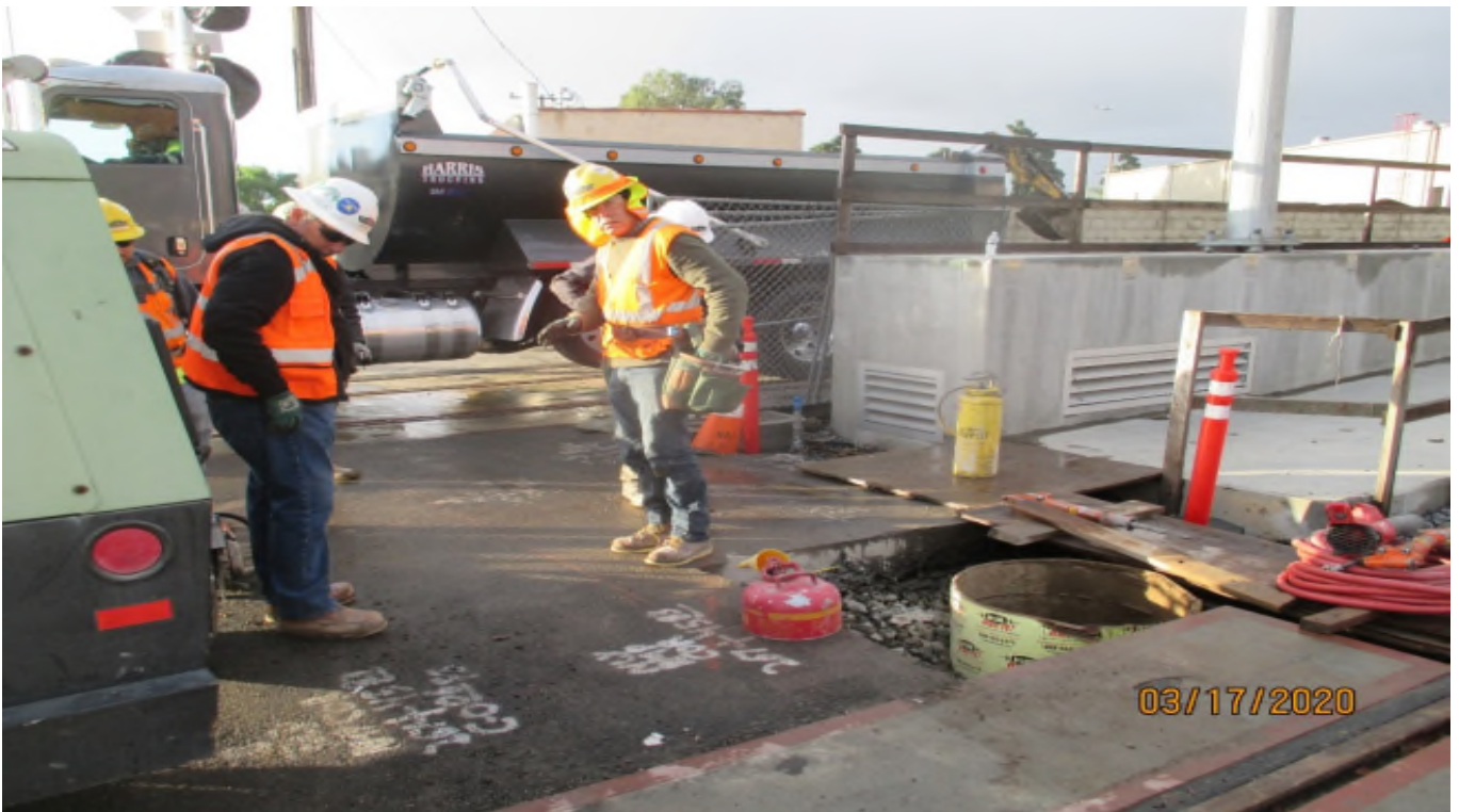
Florence/West – Layout for the Grand Pylon foundation at the east side of the West Station. Facing SW.
