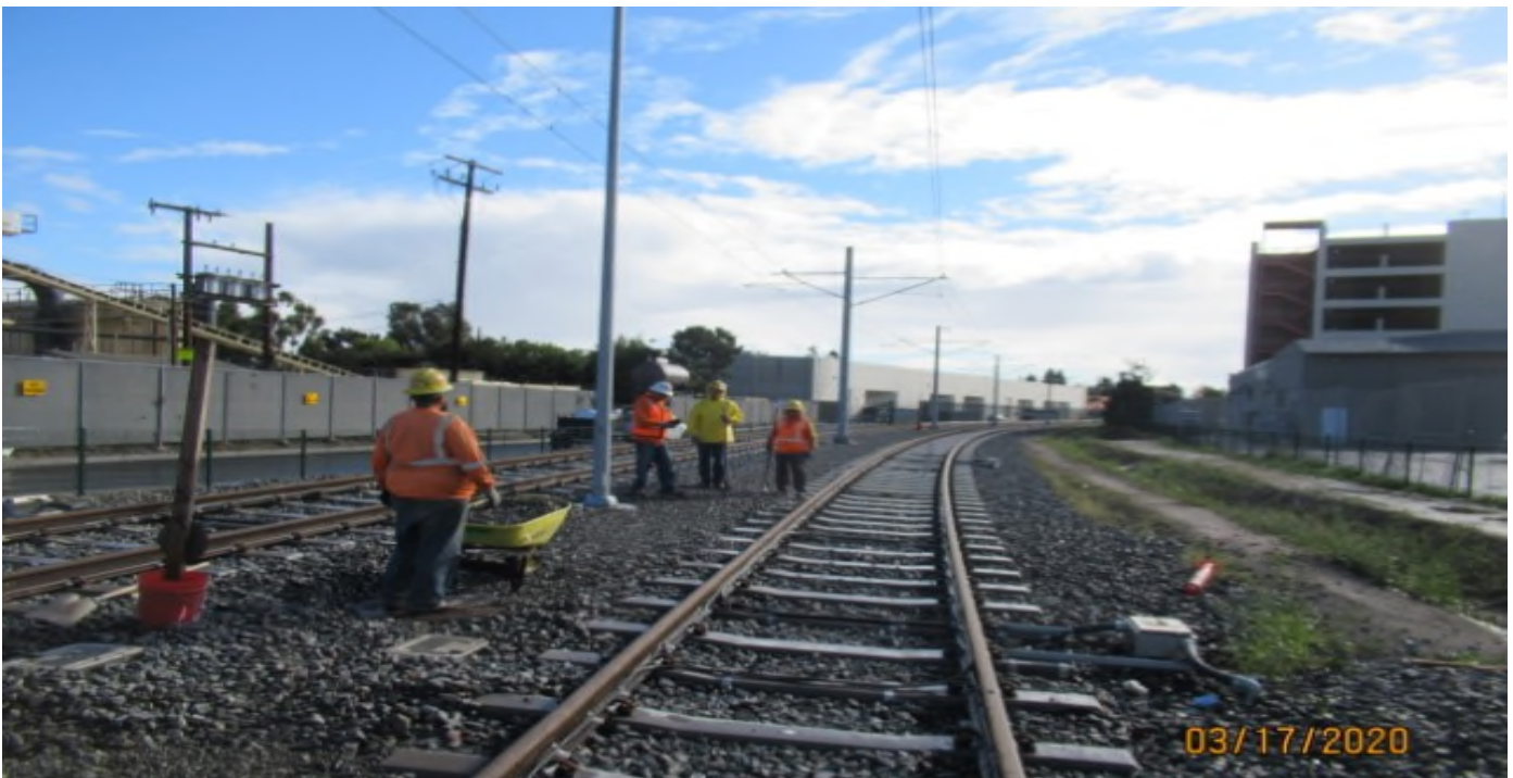
Cedar Street - WSCC Placing & dressing walkway ballast, AREMA #5 between tracks #3 & 4 north of Cedar Ave grade crossing
