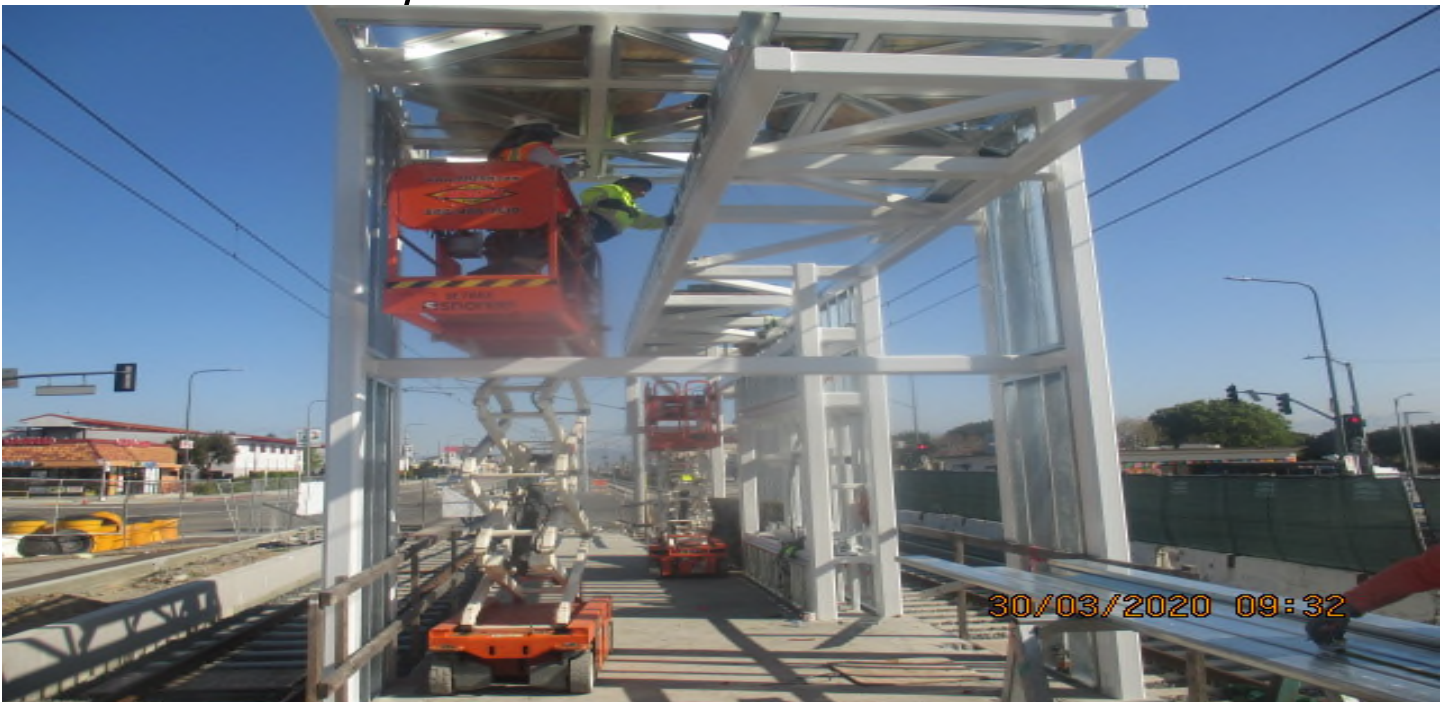
Hyde Park Station – Installing light gauge framing and roofing on the north end canopy structure. 3/30/20
