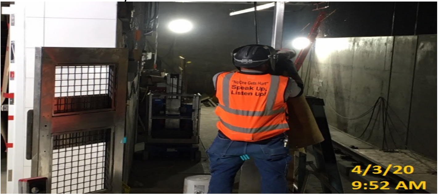
EXPO STATION – Continue end gate installation for both the north and south ends of the platform level.
