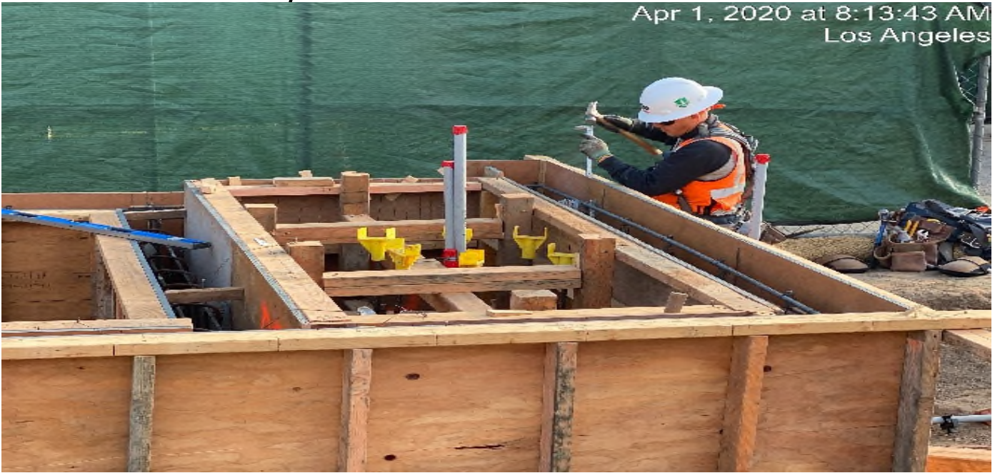
LEIMERT PARK STATION – Continue formwork for the planter wall at the east side of the plaza level.
