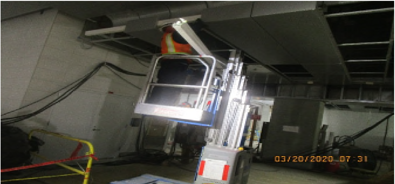
MLK STATION – Continue installing light cove and ceiling panels throughout the Free & Paid Area of the concourse level.
