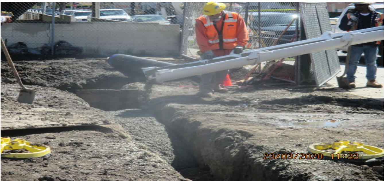
PARK MESA – Placing slurry backfill for the 12” HDPE storm drain line N-12 at TPSS#7 on 60th St & Crenshaw Blvd. 3/23/20
