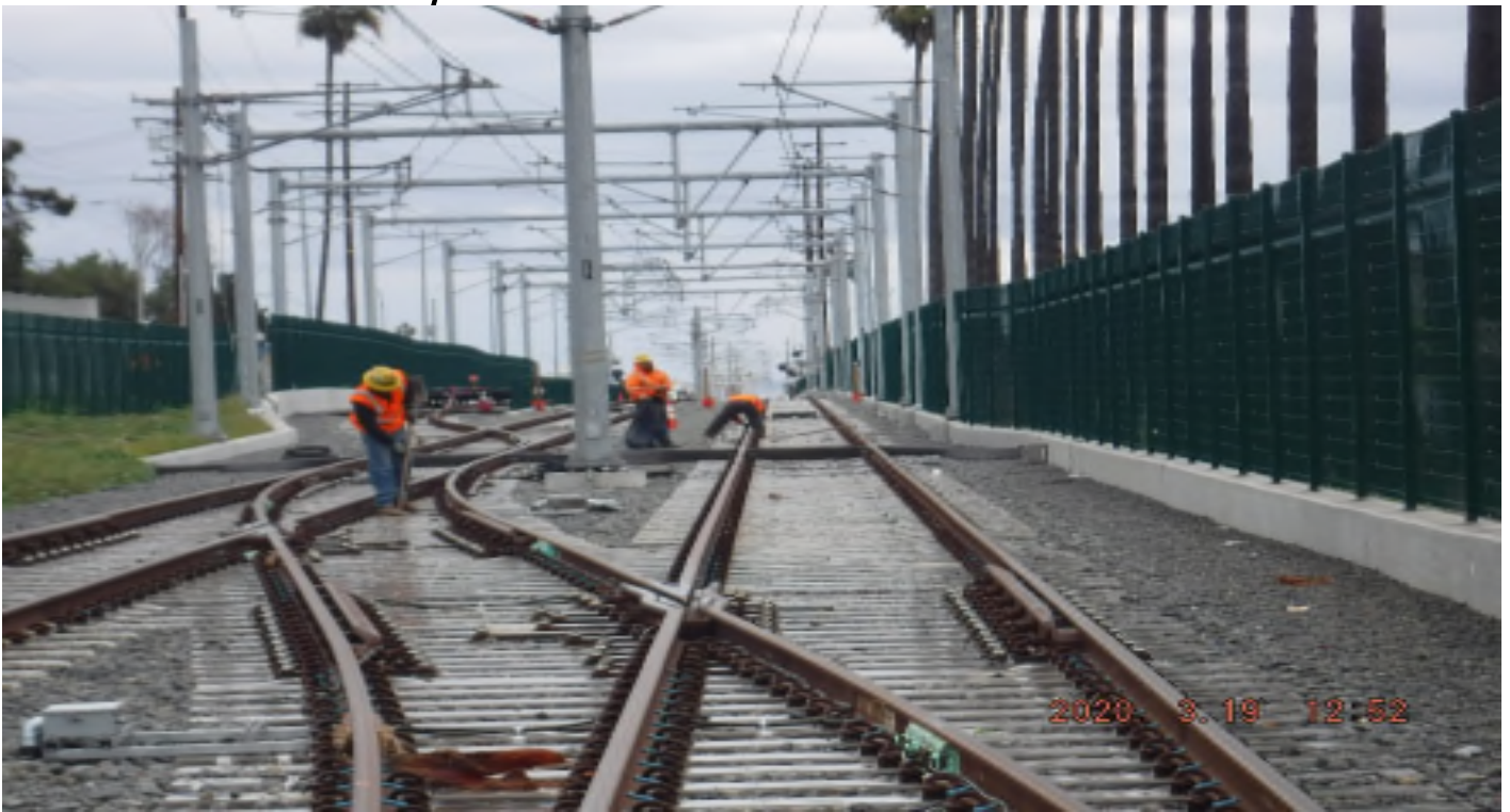
Florence/High St. - STA 245+00 TK#4 - NB looking north – track ballast cribbing and guideway housekeeping (Prairie Ave - High St)
