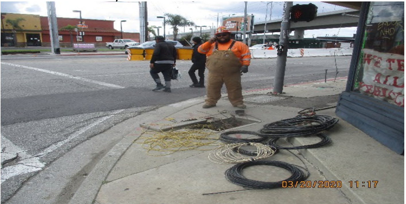
Aviation/Century – Select Electric Relocating pull boxes work at ADA ramps at intersection of Manchester and Aviation.
