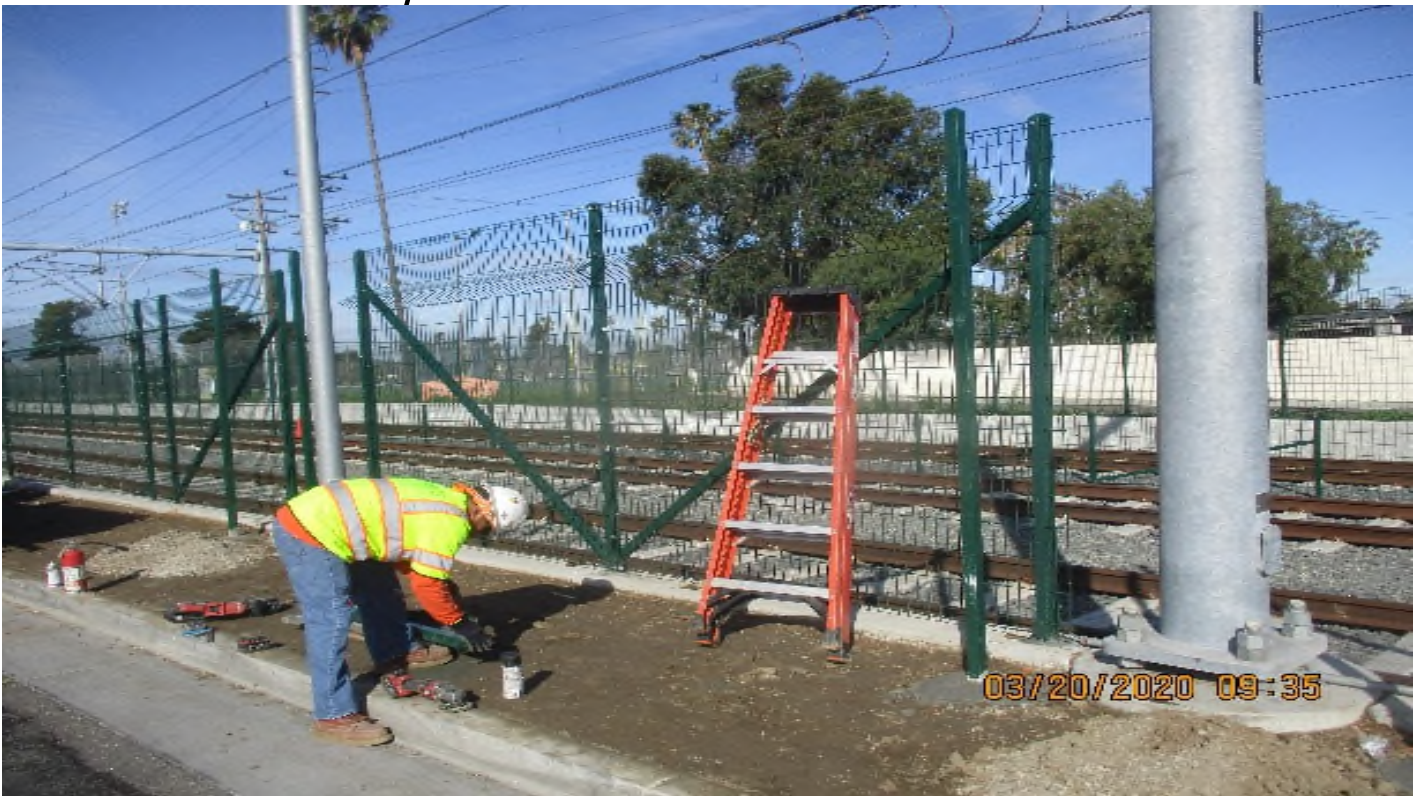
Florence/High St. - ACE Fence Place fence posts at East Bound Florence W-High
