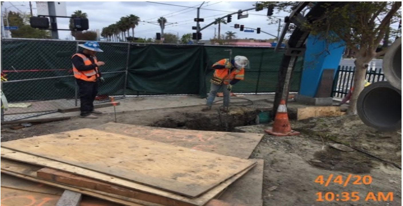
Crenshaw/Expo - EXPO – WSCC crew vacuum excavating additional depth for fiber tie in.
