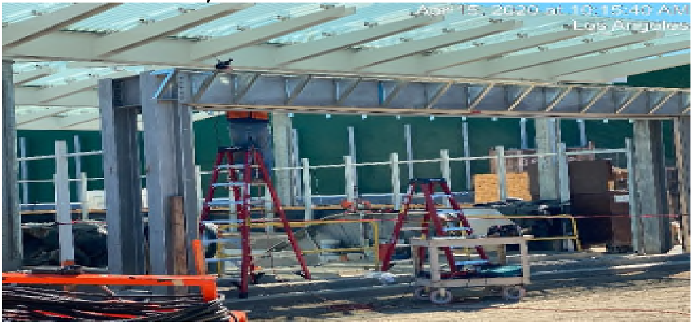
LEIMERT PARK STATION – Continue installing framing for stainless steel cladding in preparation for the overhead coiling grille installation on the main entrance canopy at the plaza level.
