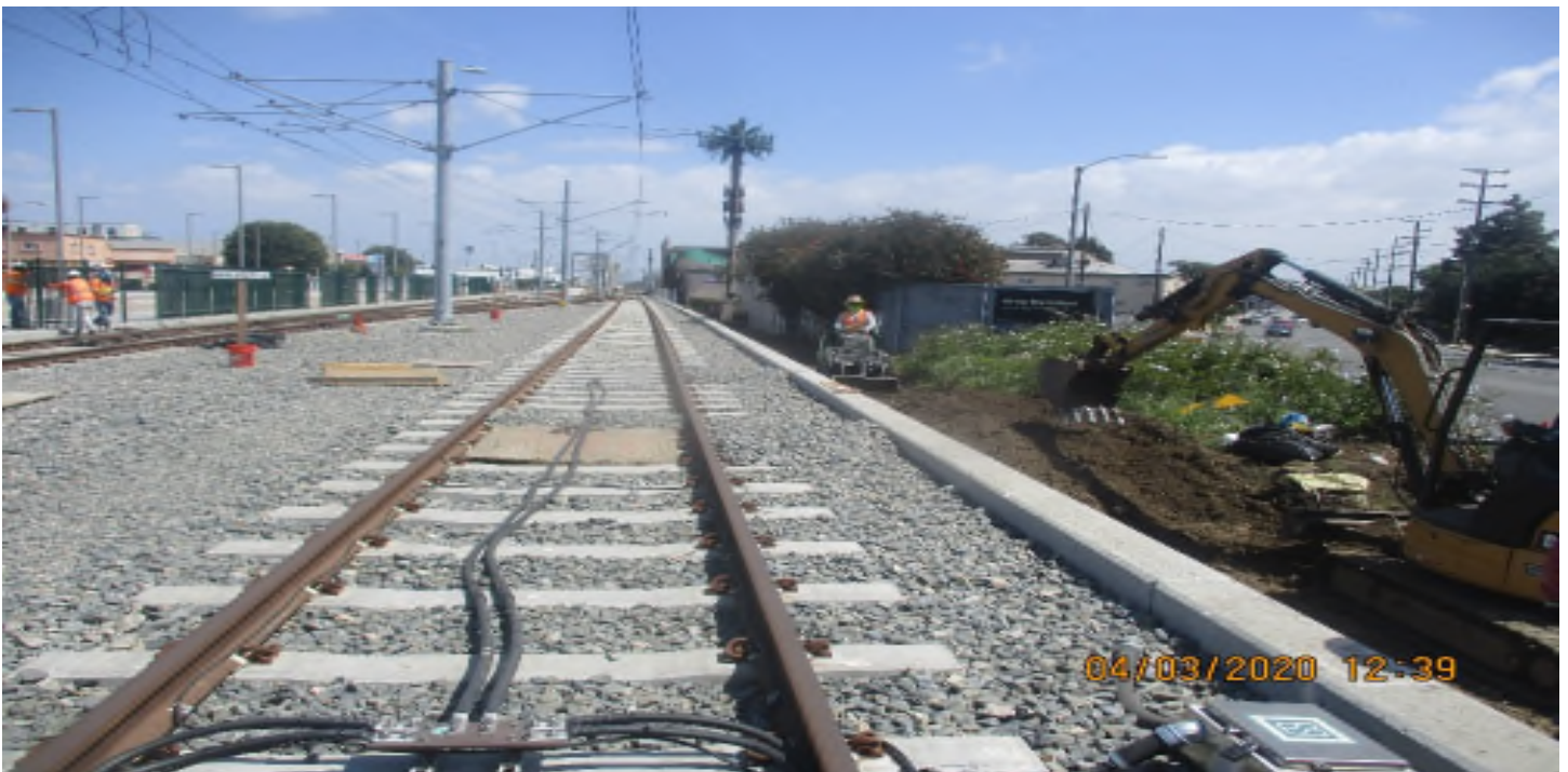
Florence/High St. - Cut slope for new swale along ballast wall east of High St.
