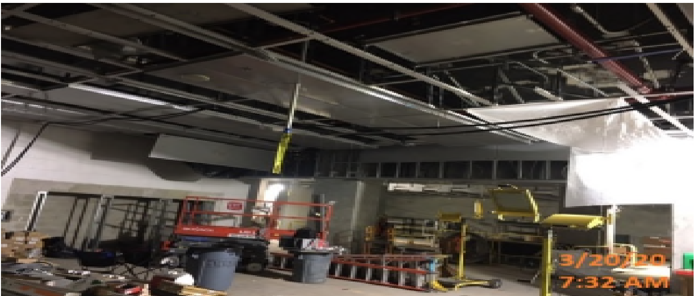
Crenshaw/Vernon - WSCC crew removing acoustic material from ceiling to investigate leak.
