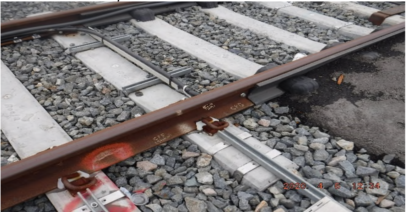
Florence/Hindry – STA 135+60 TK#4-NB looking west – right rail limit between CPF and CPG after Hindry Station platform.
