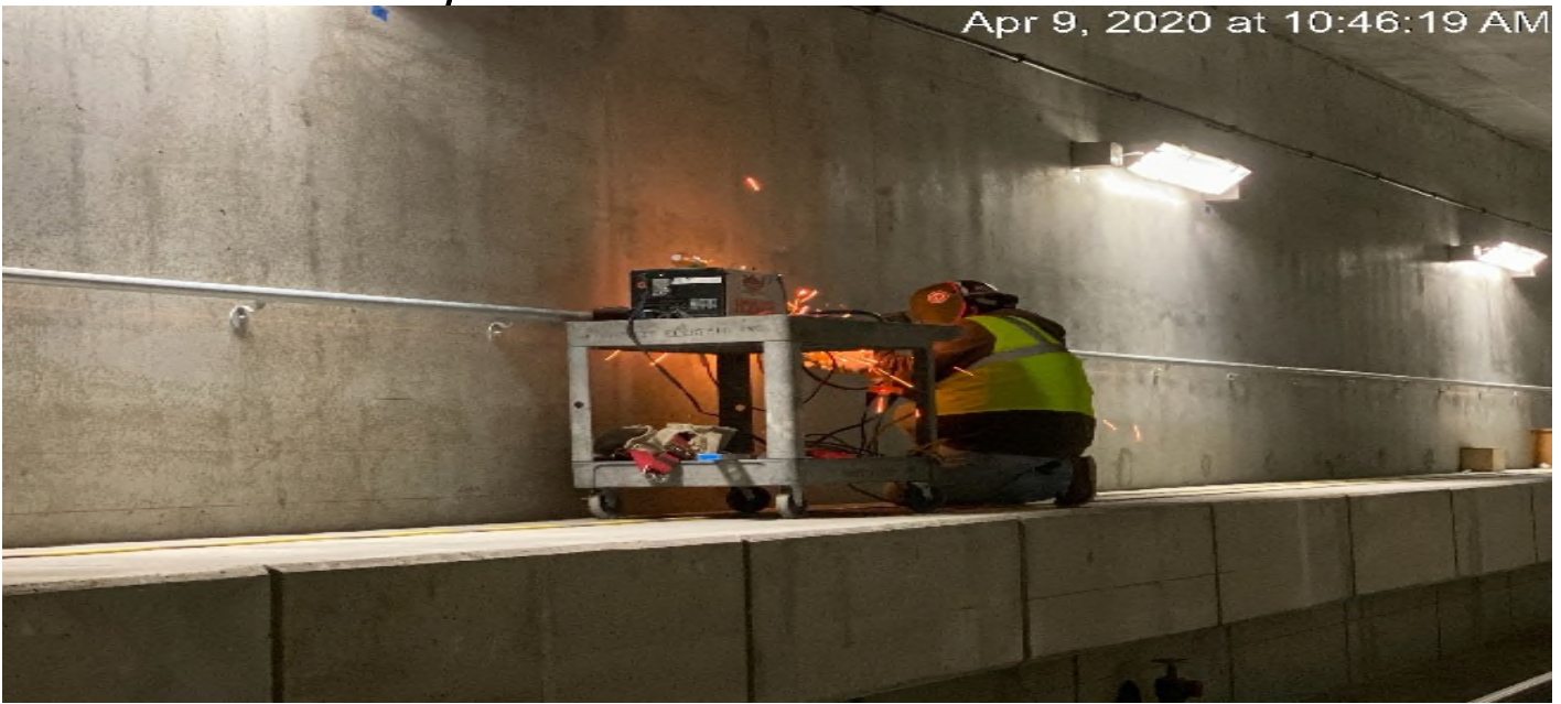
UG3 – Continue installing handrails for the emergency walkways on both the north and southbound tunnels.
