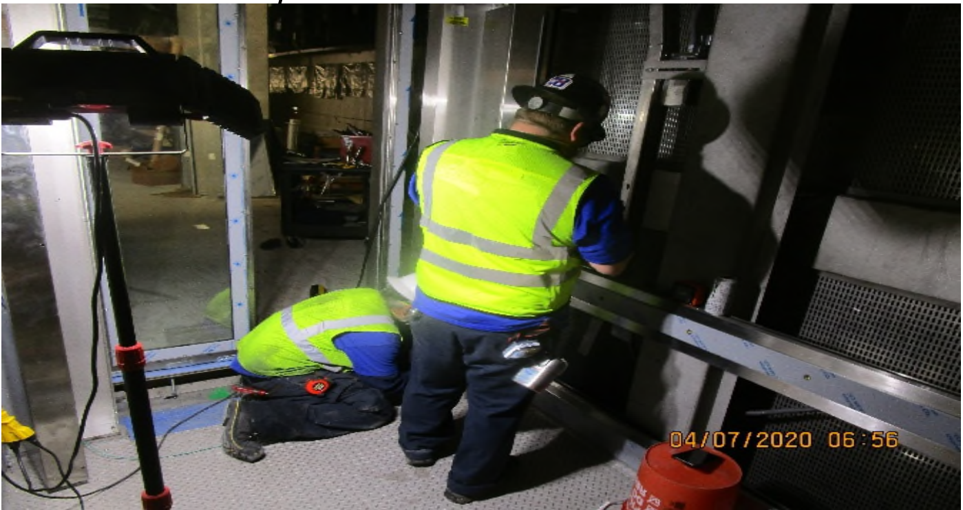
MLK STATION – Continue cab assembly and stainless steel fascia panel installation for Elevators 1&2 at the concourse level.
