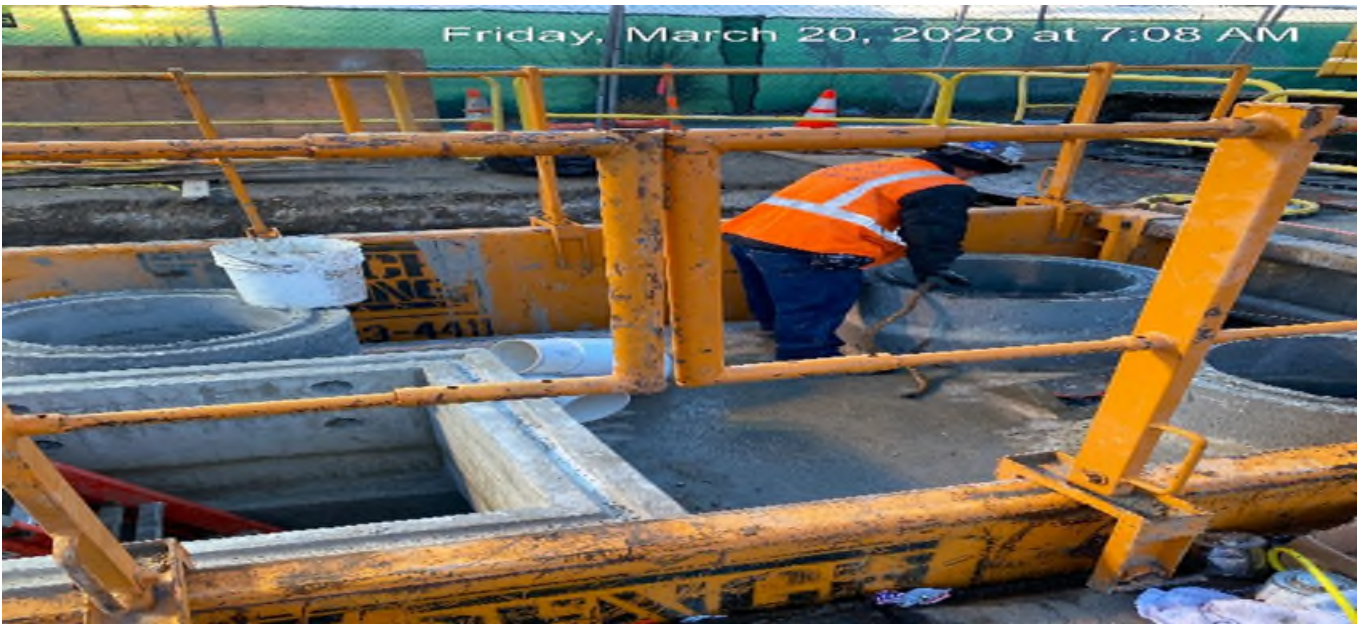
EXPO STATION – Continue oil water separator installation on Rodeo Blvd and Crenshaw Blvd.
