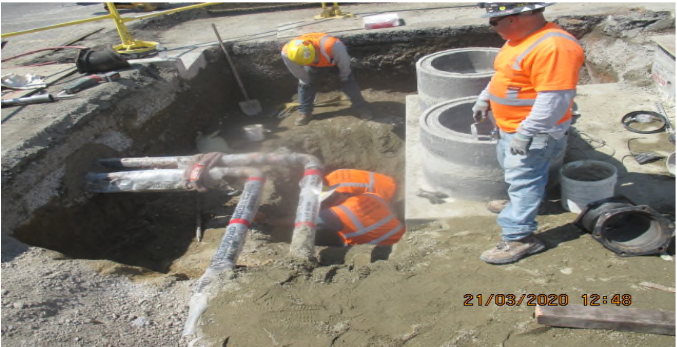
EXPO STATION – Continue oil water separator installation on Rodeo Blvd and Crenshaw Blvd.
