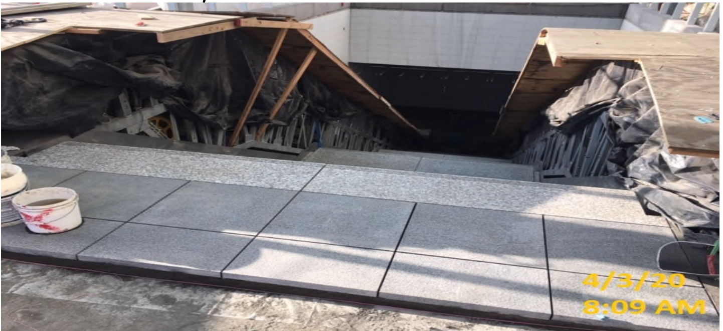
MLK STATION – Finalizing granite landing sections at the main entrance of the plaza level.
