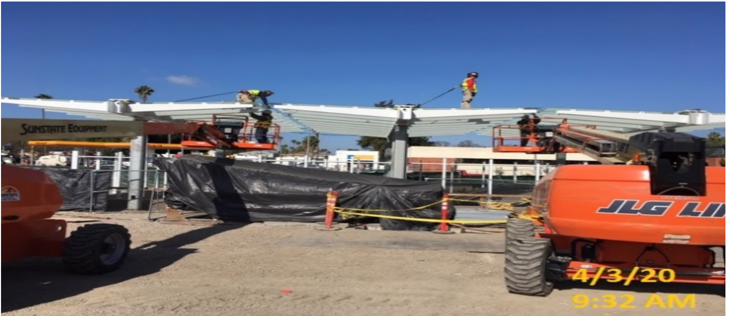
EXPO STATION – Continue tempered glass installation on top of the main entrance canopy at the plaza level.
