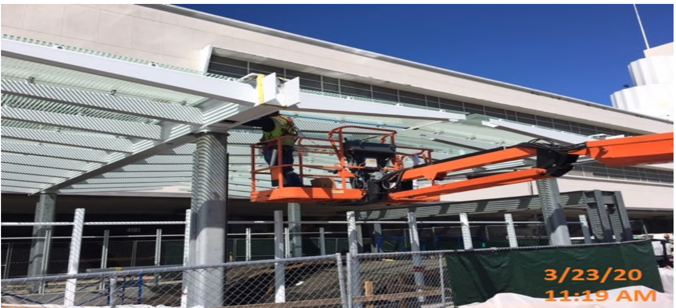
MLK STATION – Finalizing tempered glass installation above the main entrance canopy structure at the plaza level.
