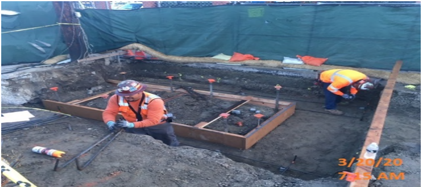
LEIMERT PARK STATION – Began formwork and placing rebar for the planter wall and footings at the west side of the plaza level.
