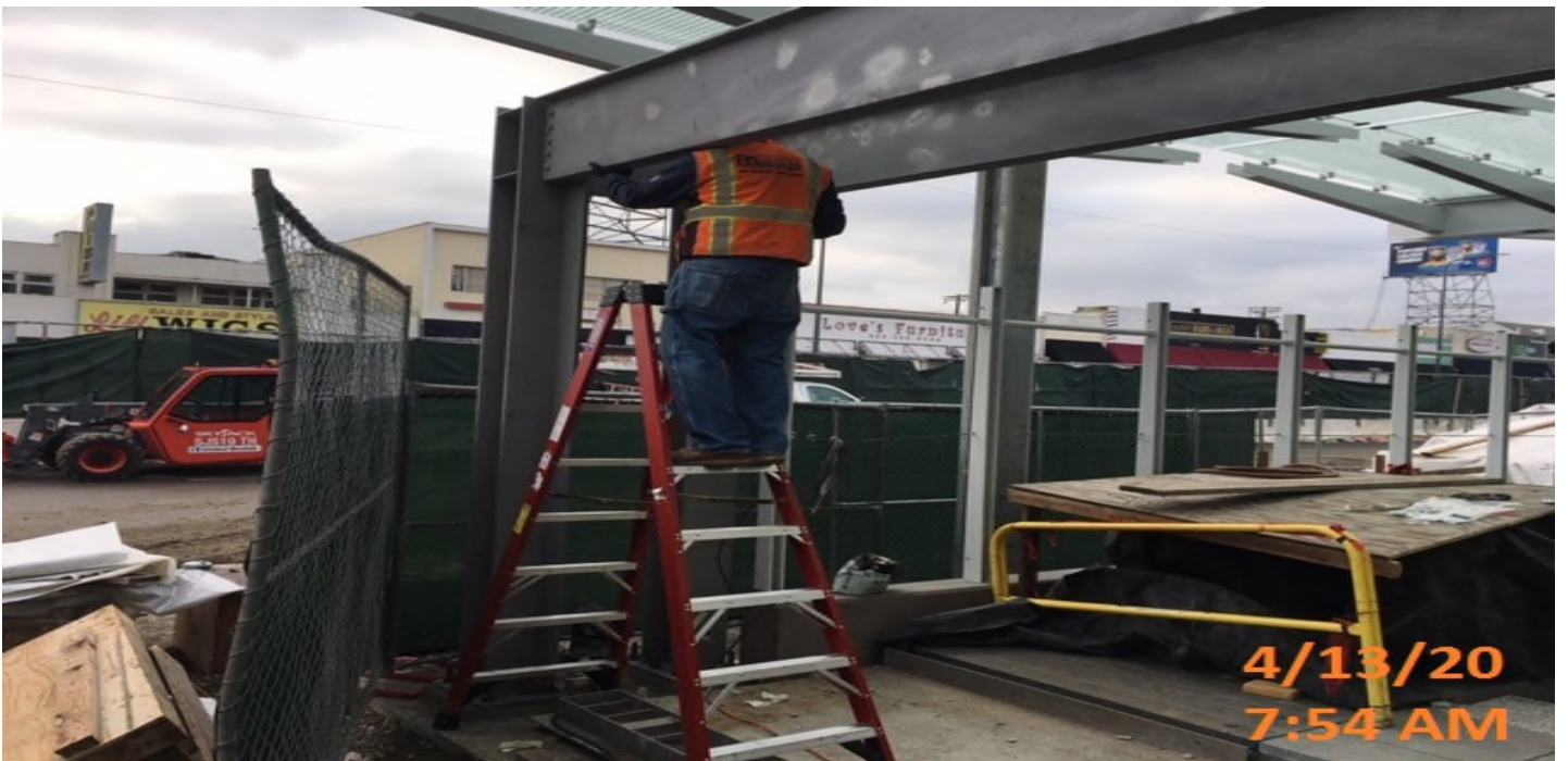
MLK STATION – Began installing overhead coiling grille components to the main entrance canopy at the plaza level.
