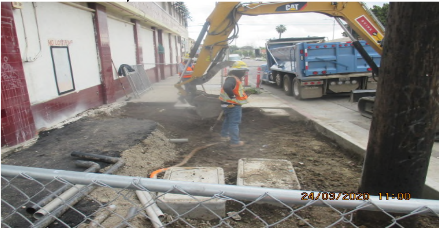
PARK MESA – Continue excavating for new sidewalk and ADA ramp installation on the northeast corner of 54th St and Crenshaw Blvd. 3/24/20
