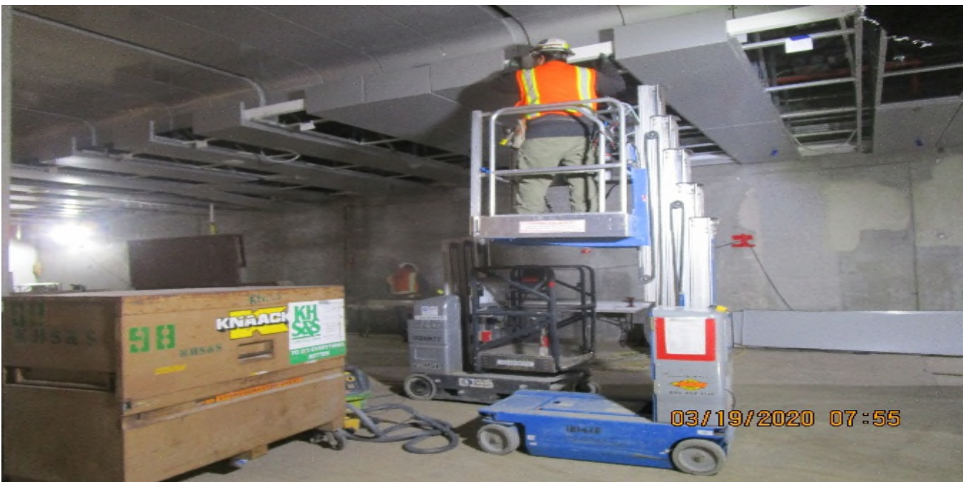
MLK STATION – Continue installing light cove and ceiling panels throughout the Free & Paid Area of the concourse level.
