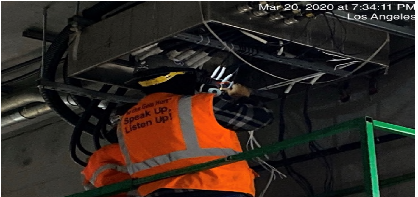
UG3 – Continue splicing wires for the tunnel booster junction boxes at the southbound tunnel at Sta 291+50.
