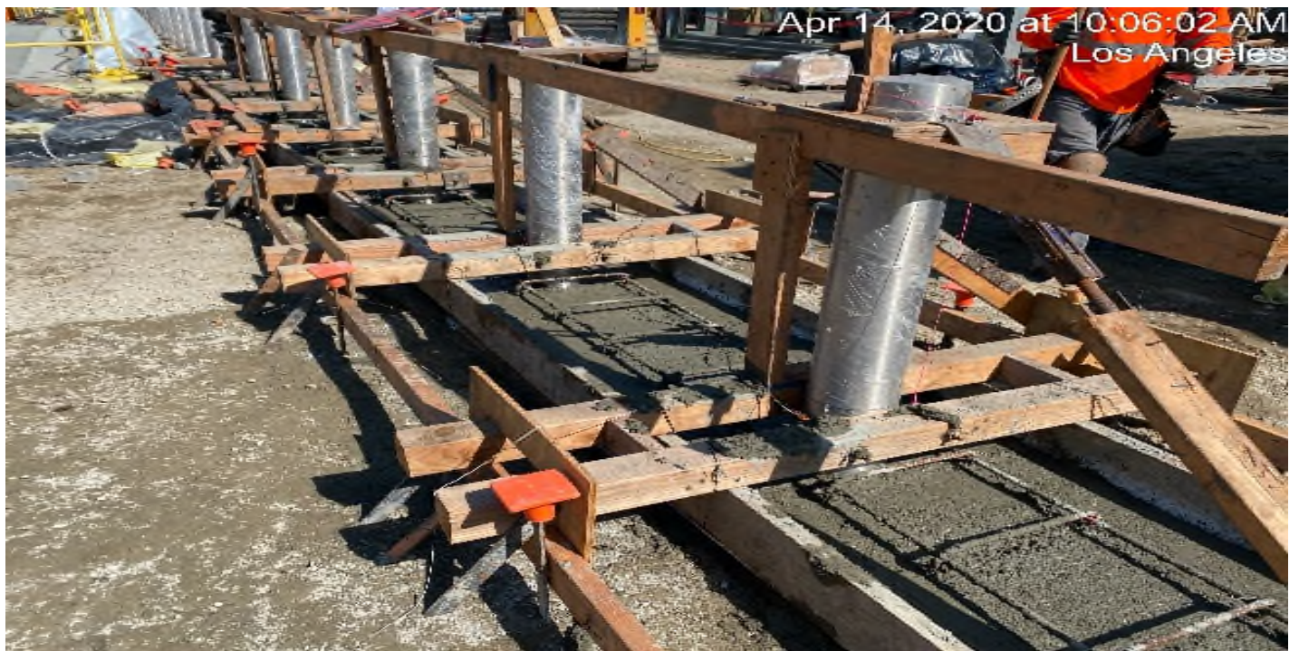
LEIMERT PARK STATION – Placing concrete for the stainless steel bollards at the plaza level.
