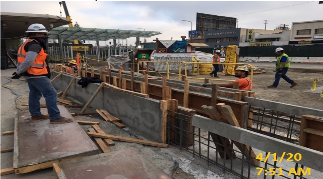
Crenshaw/MLK - MLK – WSCC crew stripping and building formwork for west planter wall.
