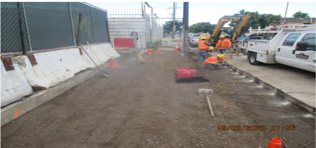
UG3 – Continue grading/compaction for the new sidewalk/driveway installation on the southwest corner of 67th St and Crenshaw Blvd. 3/18/20
