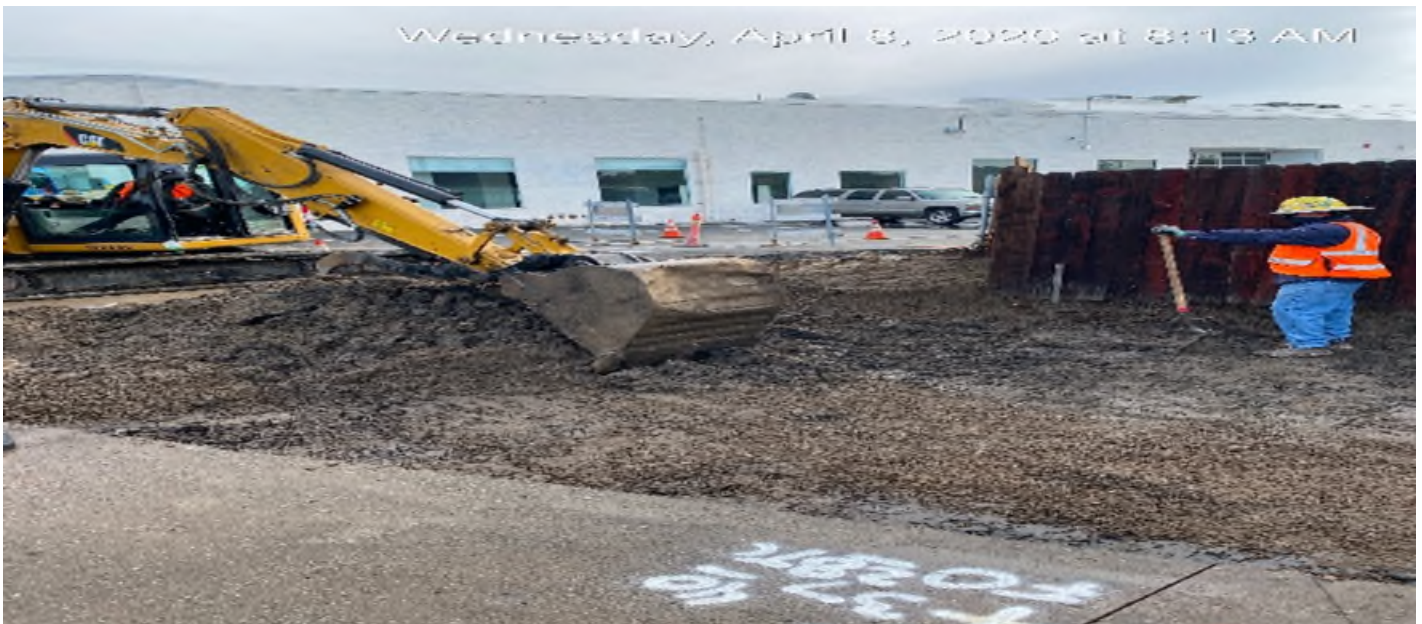
EXPO STATION – Continue excavating for new sidewalk and ADA ramp installation on Bronson Ave east of the plaza.
