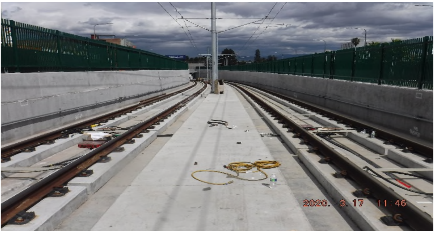
48 th Street - STA 365+00 looking north – Train Control (TC) system work south ramp of UG4, 48th St behind camera.
