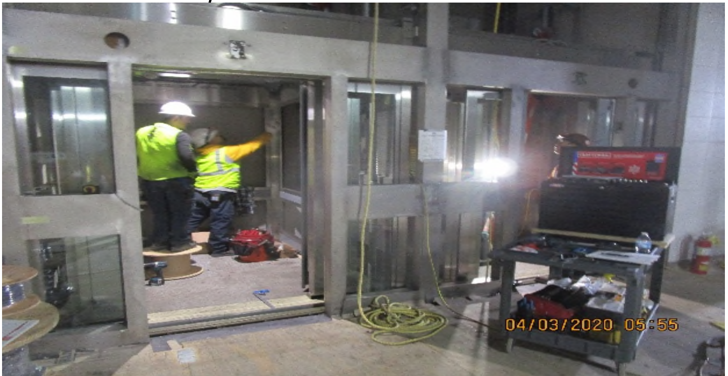
Crenshaw/Vernon - Vernon Concourse, Elevators 3, begin re-work of hoist way electrical conduit that is encroaching into hoist way.
