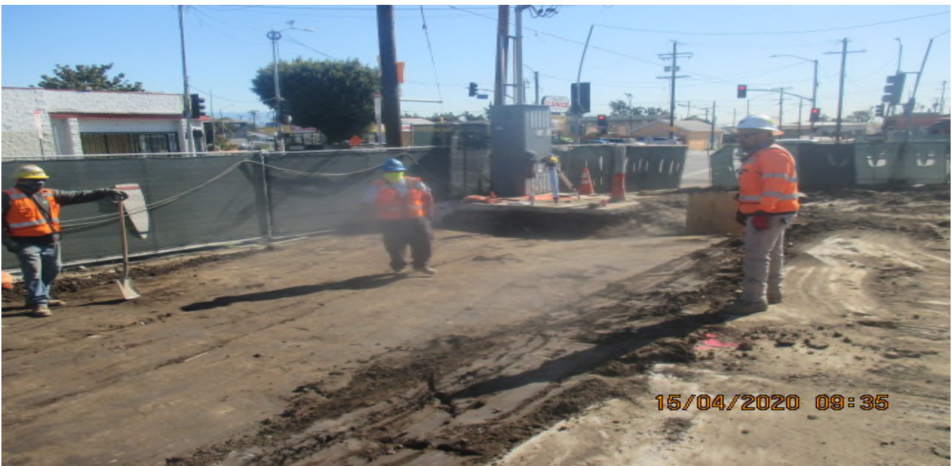
UG3 – Continue grading and excavating for the culvert drainage along the eastbound sidewalk of 67th St in preparation for concrete placement. 4/15/20
