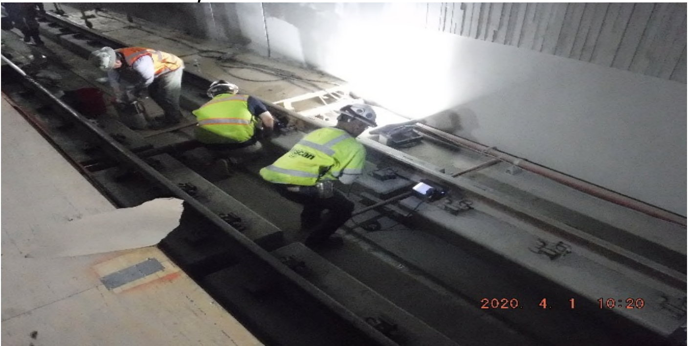
Crenshaw/Expo - STA 448+00 TK#4-NB looking north – plinth rebar scanning in progress UG4 Exposition Station.
