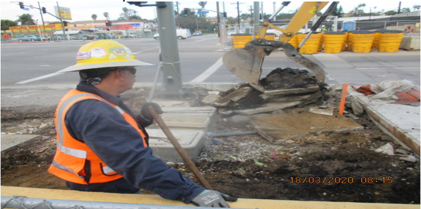
PARK MESA – Continue excavating/demolishing for new concrete sidewalk installation on the northeast corner of 48th St and Crenshaw Blvd. 3/18/20
