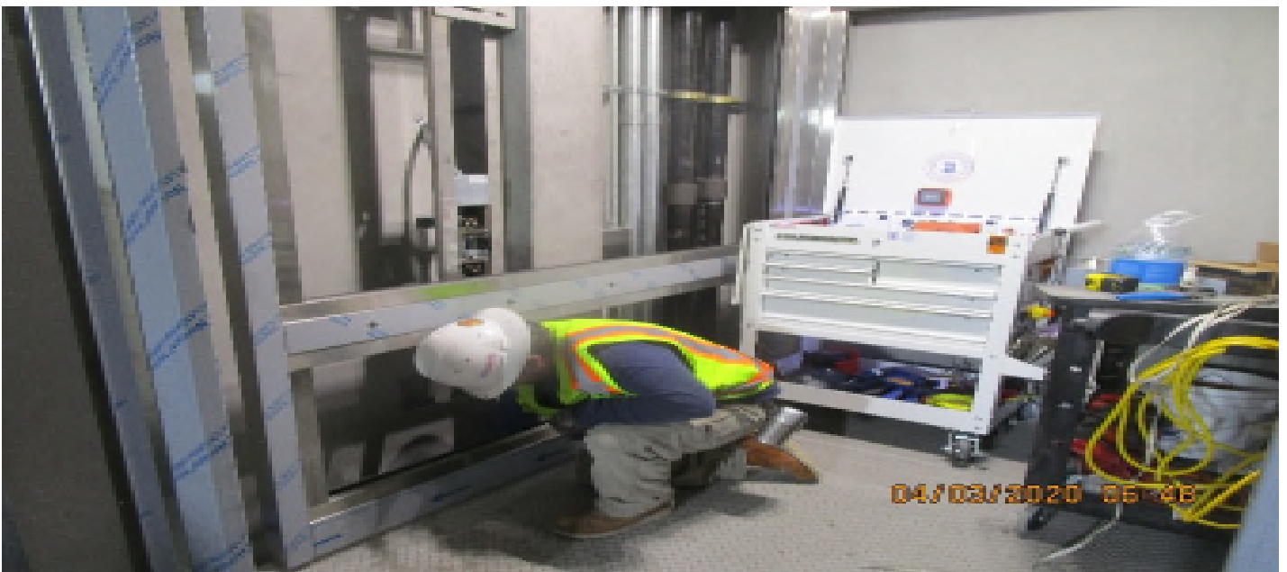
MLK STATION – Continue cab assembly and stainless steel fascia panel installation for Elevators 3&4 at the concourse level.
