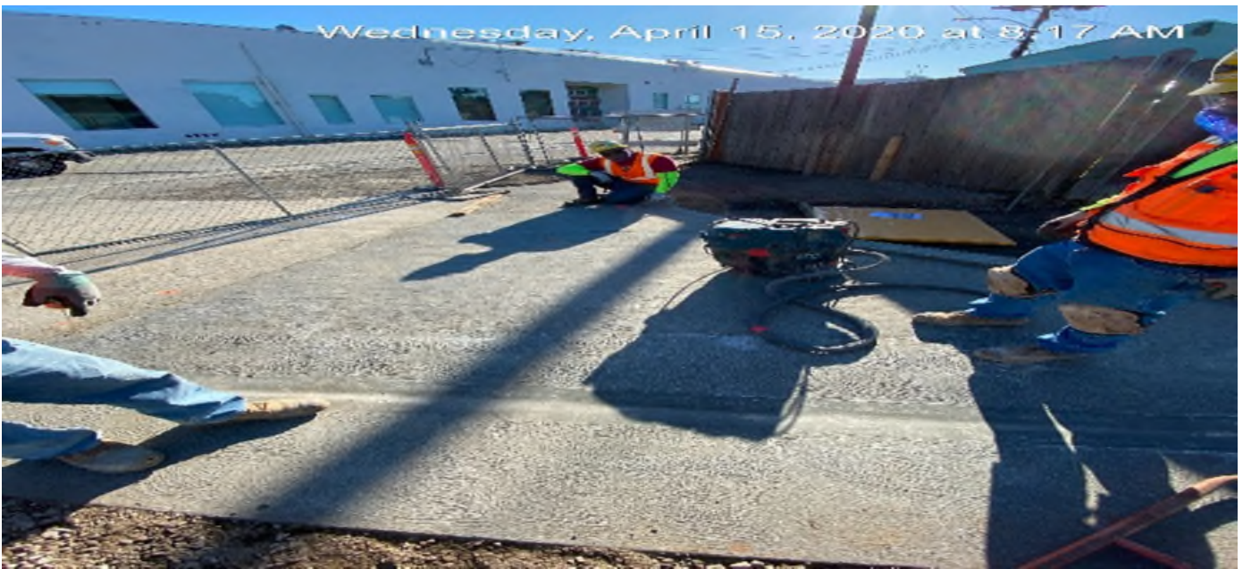
EXPO STATION – Began saw cutting the sidewalk concrete on Bronson Ave east of the plaza.
