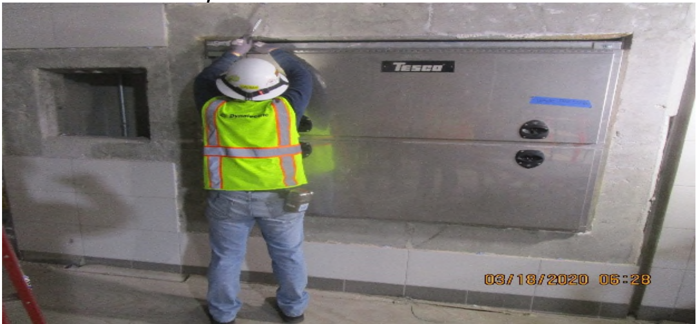
LEIMERT PARK STATION – Resume emergency management panel installation at the concourse level.
