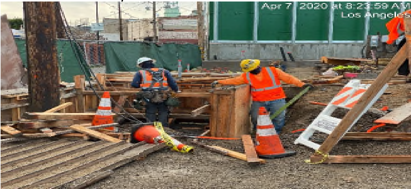
LEIMERT PARK STATION – Continue working on the planar wall installation at the east side of the plaza level.
