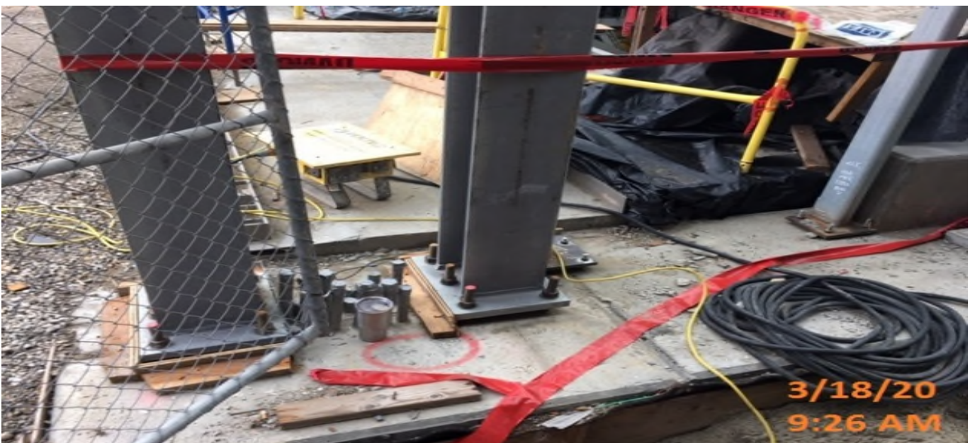
MLK STATION – Continue building forms for the metal base plates of the main entrance canopy columns at the plaza level.
