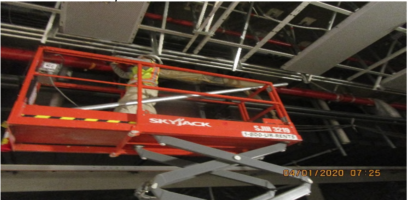
Crenshaw/MLK - MLK Platform, Continued rough in 2" GRC for Radiax & coaxial cable support W-O benefit of AFC drawings.
