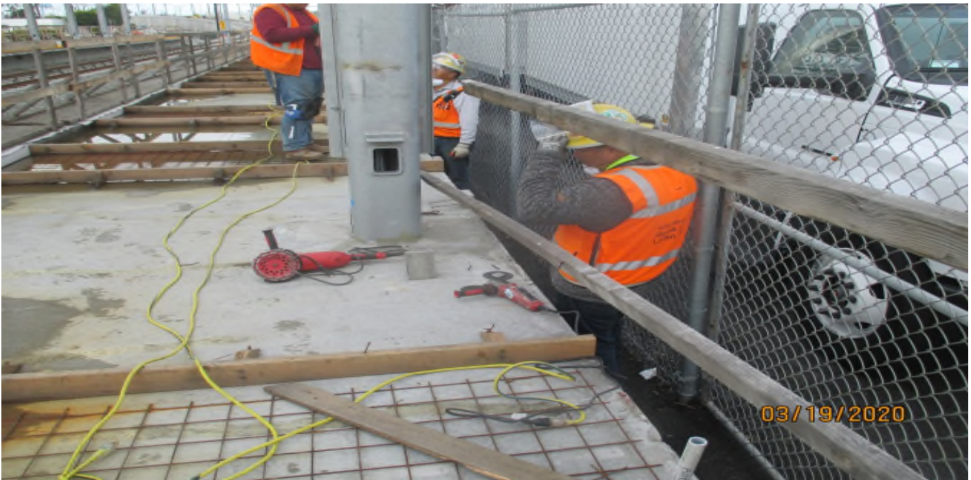
Florence/Hindry – Removal of the fence post mounts at the Hindry Station SB platform.
