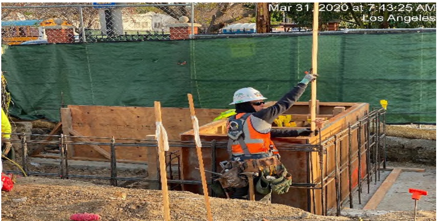
LEIMERT PARK STATION – Continue formwork for the planar wall at the east side of the plaza level.
