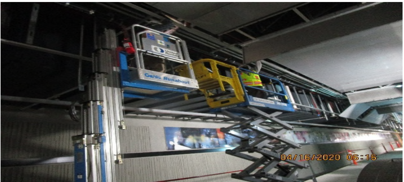
LEIMERT PARK STATION – Continue radiax cable conduit and support rack installation on the platform ceiling level.
