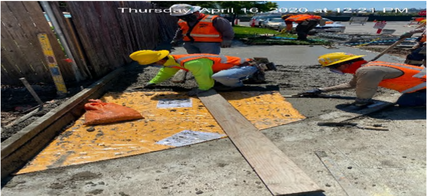
EXPO STATION – Placing concrete for the new ADA ramp installation on Bronson Ave east of the plaza.
