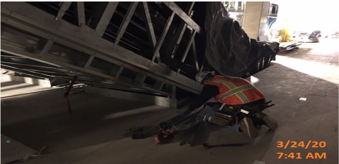
MLK STATION – Continue installing steel stud track and framing underneath escalator 3 at the platform level.
