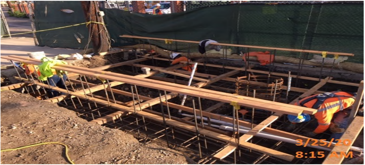
LEIMERT PARK STATION – Continue formwork and placing rebar for the planar wall and footings at the east side of the plaza level.
