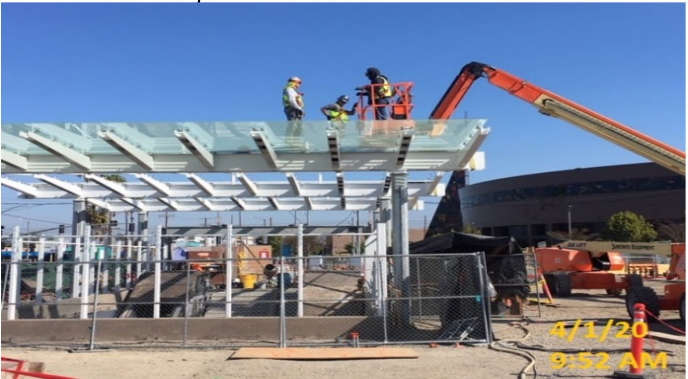
Crenshaw/Expo - EXPO – Giroux Glass installing glass panels at main entrance canopy platform end gates.
