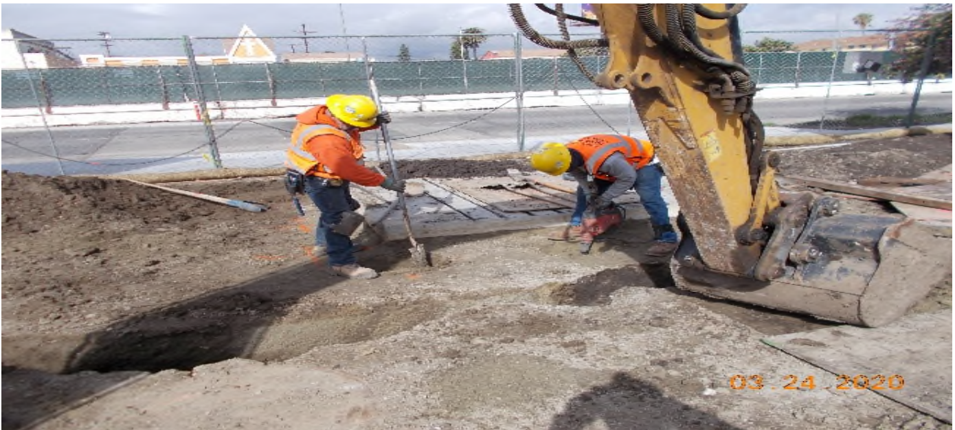
PARK MESA – Excavating for bollard installation around the DWP transformer pad at TPSS#7 on 60th St & Crenshaw Blvd.
