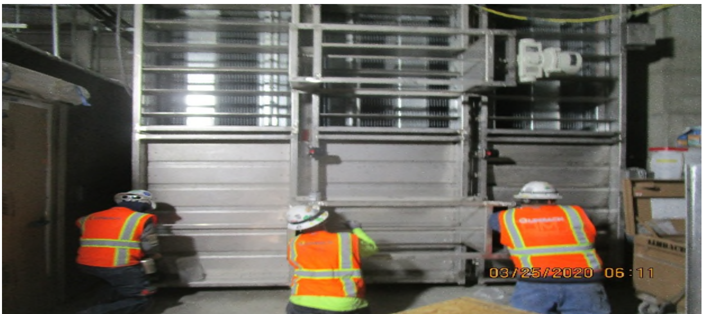
LEIMERT PARK STATION – Continue tunnel fan damper section installation for the sound attenuator for EVF-6-302 in the North Fan Room C – 142 of the concourse level.
