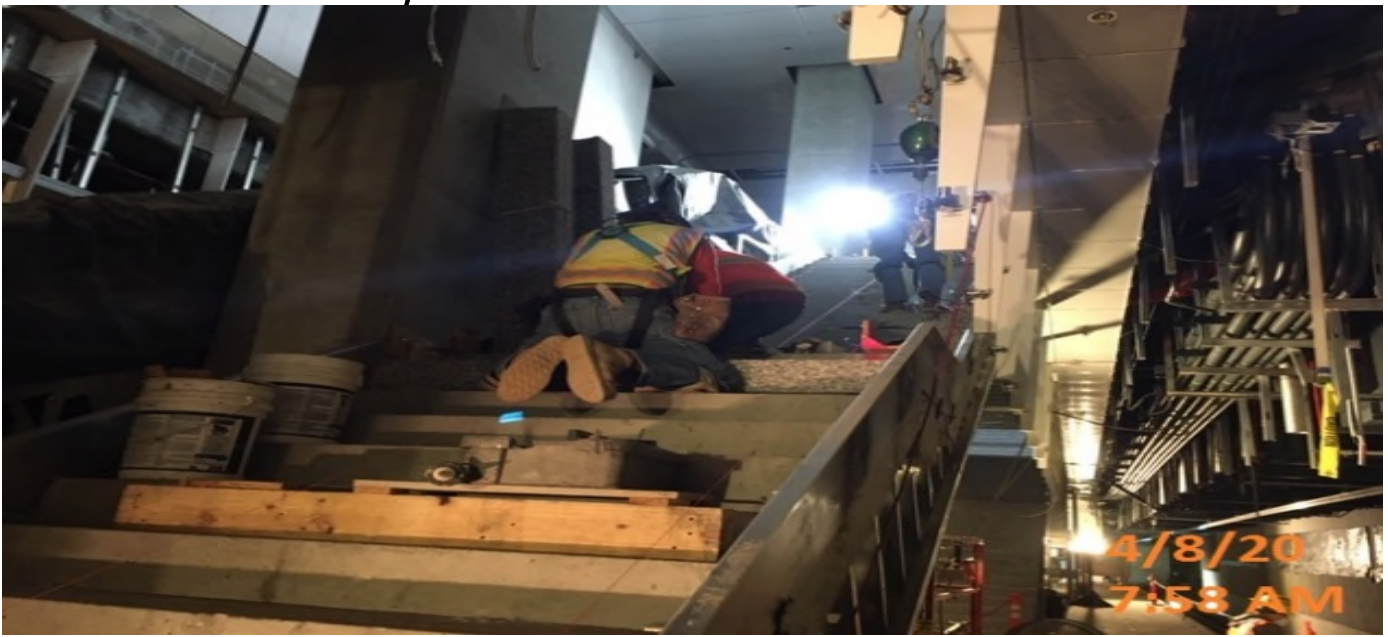
MLK STATION – Continue installing granite treads and landing sections for staircases 2&3 between concourse and platform level.
