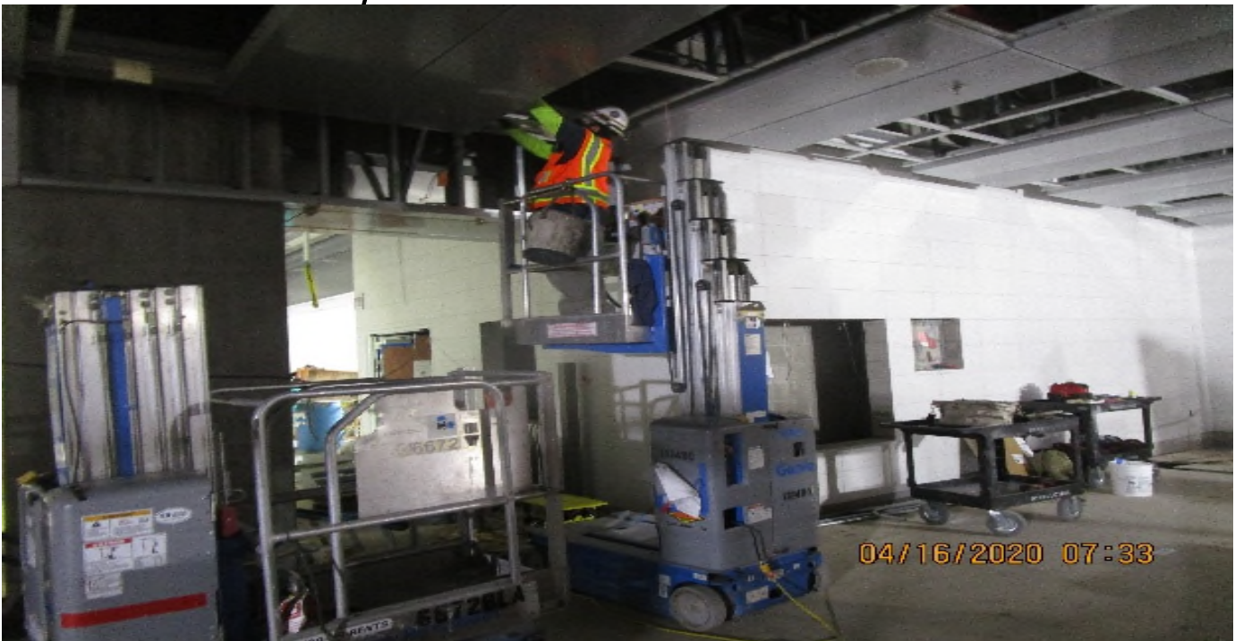
MLK STATION – Installing flex whips for the drop ceiling light fixtures at the concourse level.
