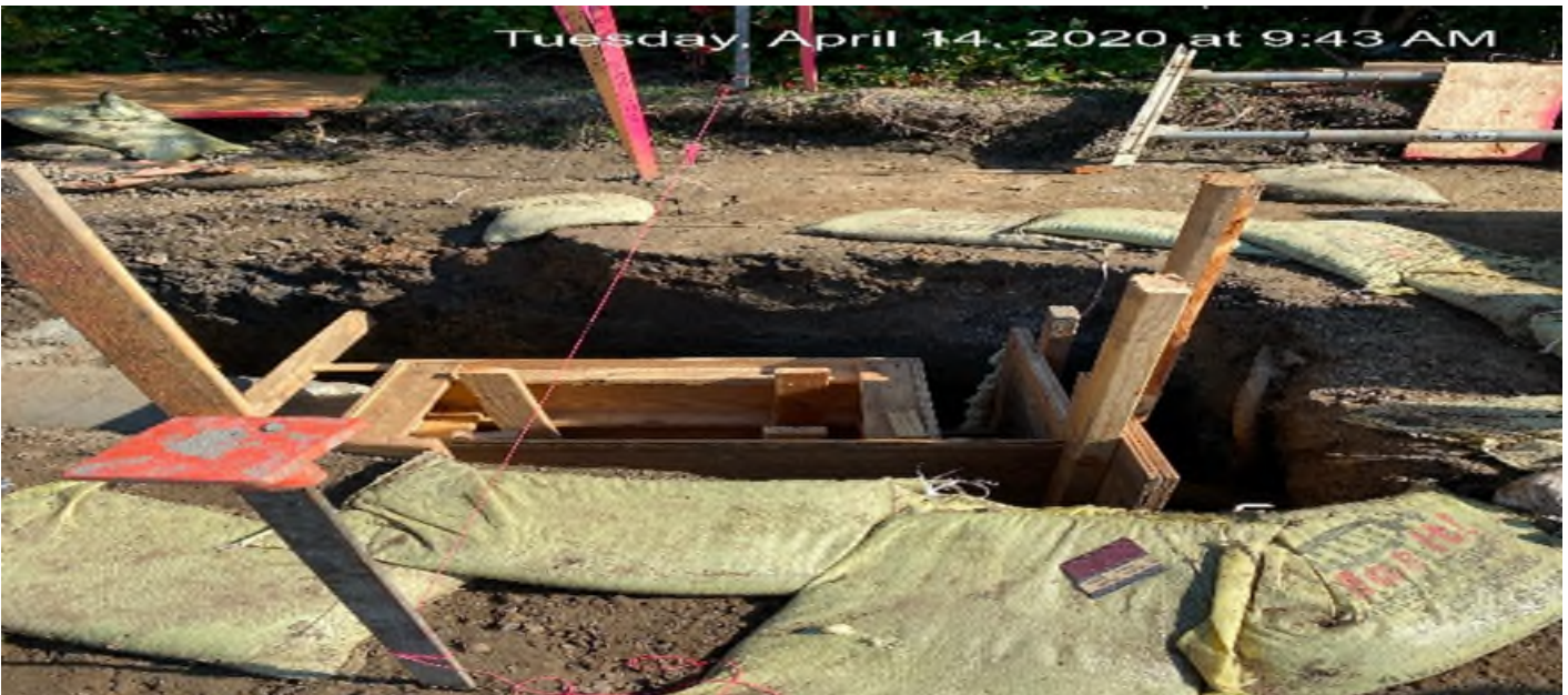
EXPO STATION – Forming Catch Basin #2 in preparation of concrete placement on the northwest section of the plaza.
