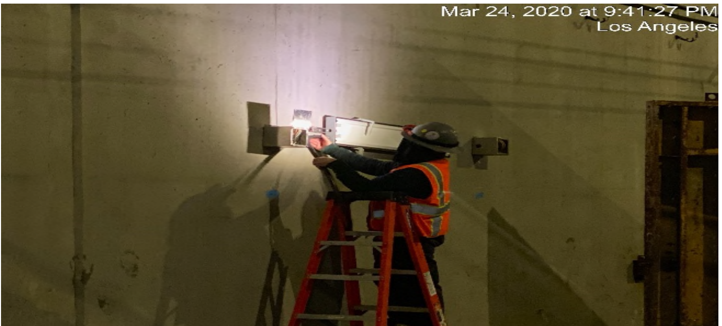
UG3 – Continue pulling wire for the emergency lighting on the northbound tunnel of the south end portal entrance.
