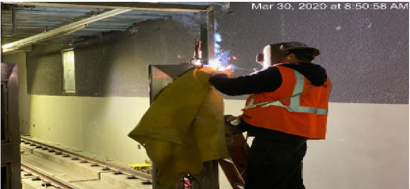
LEIMERT PARK STATION – Continue end gate installation for both the north and south end of the platform level.
