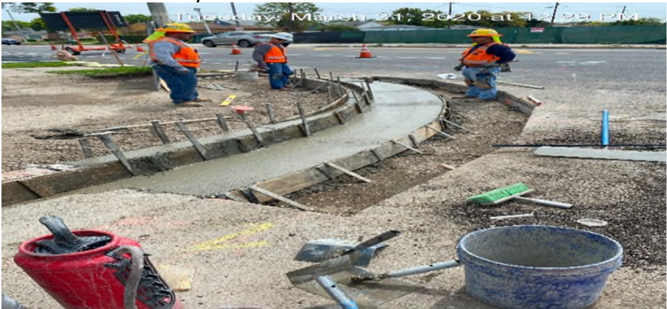
EXPO STATION – Building forms and placing concrete for new curb/gutter and ADA ramp installation on Bronson Ave east of the plaza.
