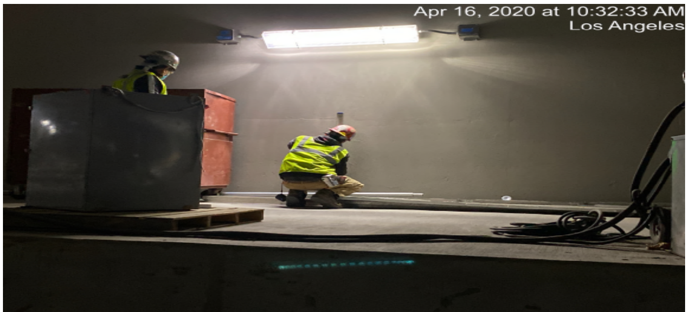
UG4 – Continue handrail installation for the emergency walkways along the southbound tunnel.
