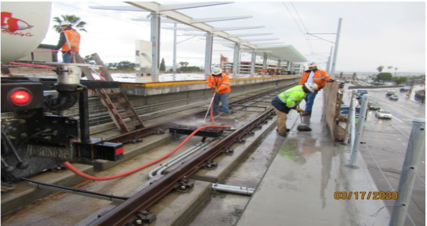
Aviation/Century – HCC at Century Aviation station platform cleaning guideway with high pressure water truck.
