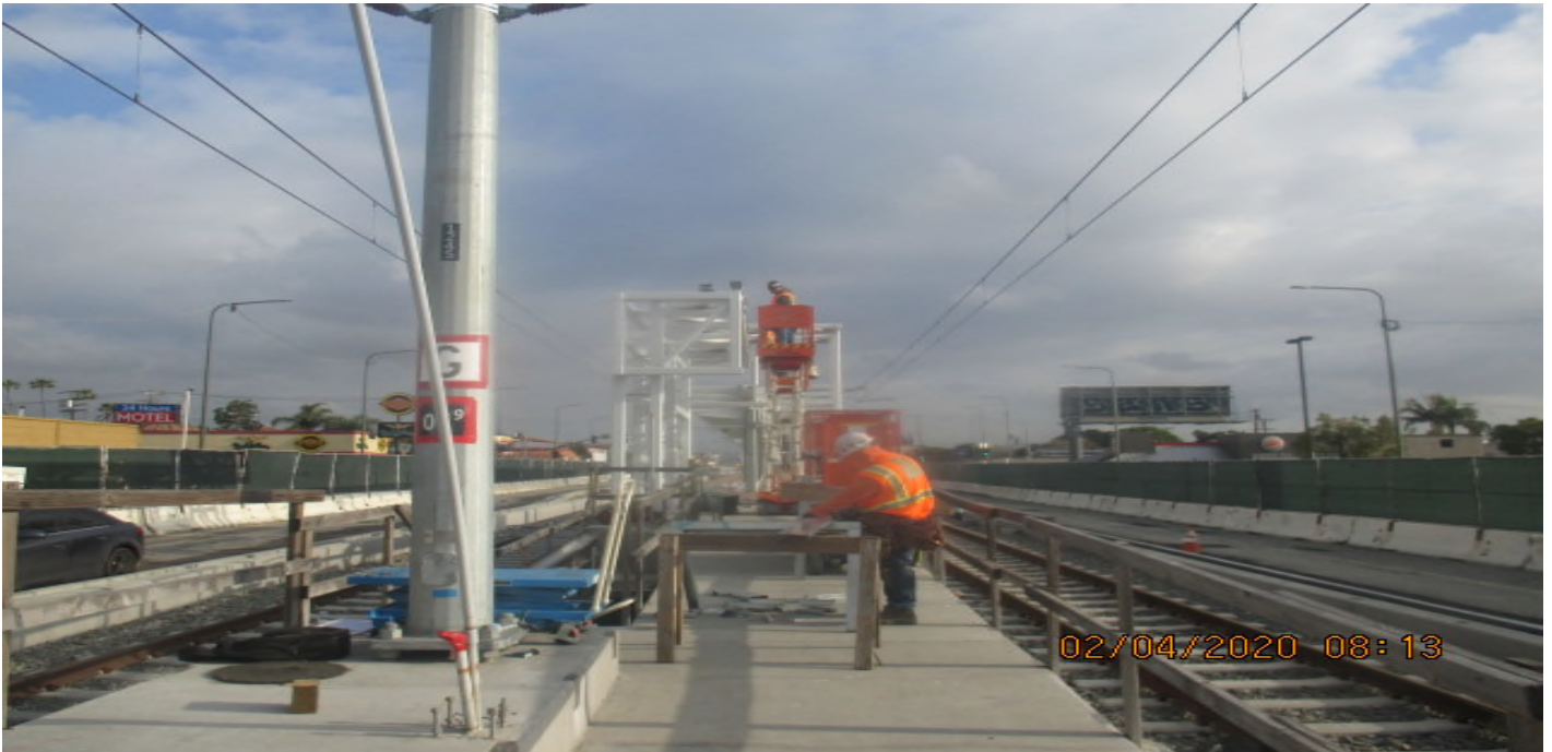
Hyde Park Station – Continue installing light gauge framing and roofing on the south end canopy structure. 4/2/20
