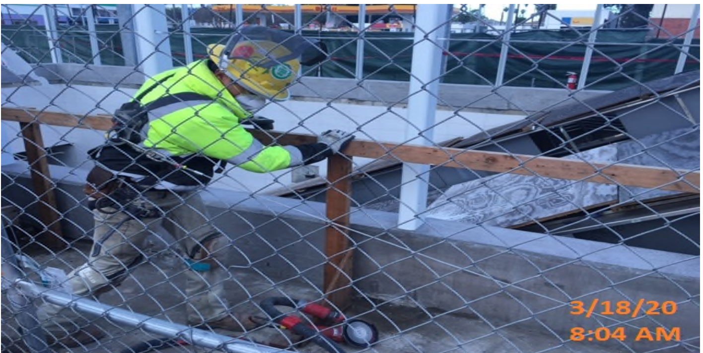
EXPO STATION – Continue surface finishing the wind screen curbs around the main entrance of the plaza level.
