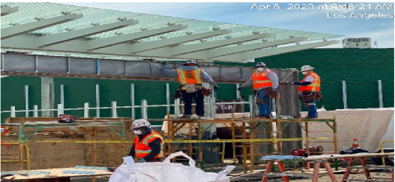
LEIMERT PARK STATION – Installing framing for stainless steel cladding in preparation for the overhead coiling grille installation on the main entrance canopy at the plaza level.
