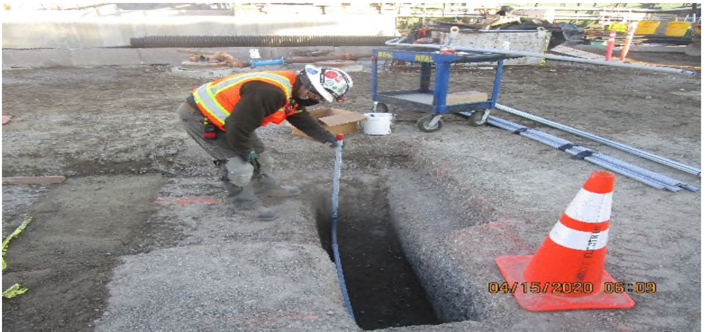
Crenshaw/Vernon - Plaza level, North of Station entrance begin rough in 1" PVC to footing of free-standing map case.
