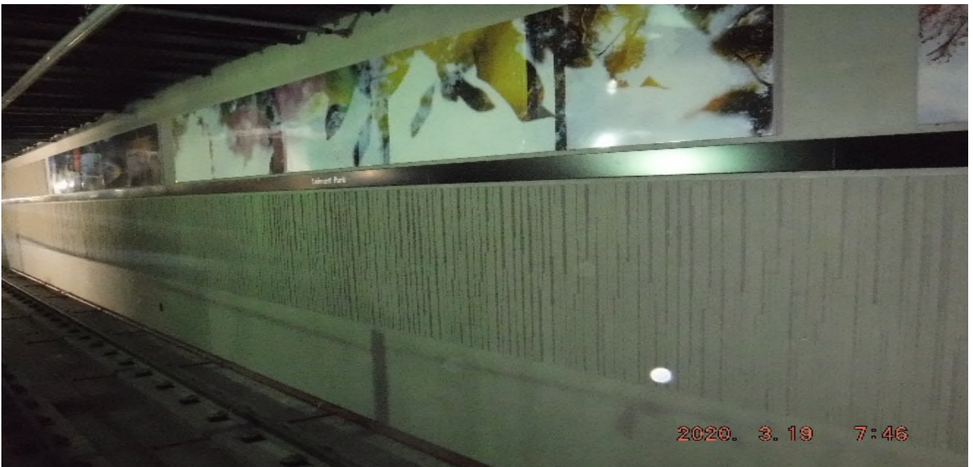
Florence/West – STA 267+40 TK#3 - SB looking north – vacuum fine materials from track ballast (West)
