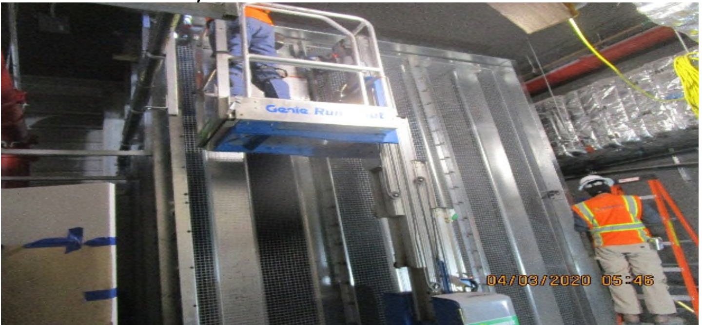
Crenshaw/Vernon - Emergency fan room (S) continued rough in & bolting bird screens prep to install TFD-6-301 per RFI-029.
