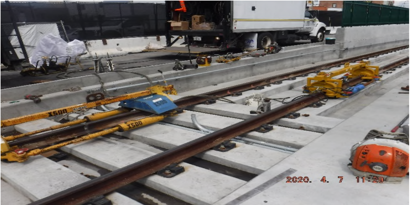
48 th Street - STA 364+70 TK#3-SB looking north – rail de-stress in progress (48th St behind camera).
