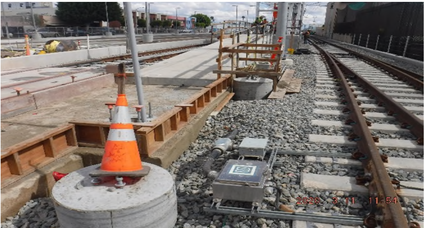
Florence/West – track ballast partly backfilled around new light pole foundation w.o control of sub-ballast refurbishing – PUNCH LIST
