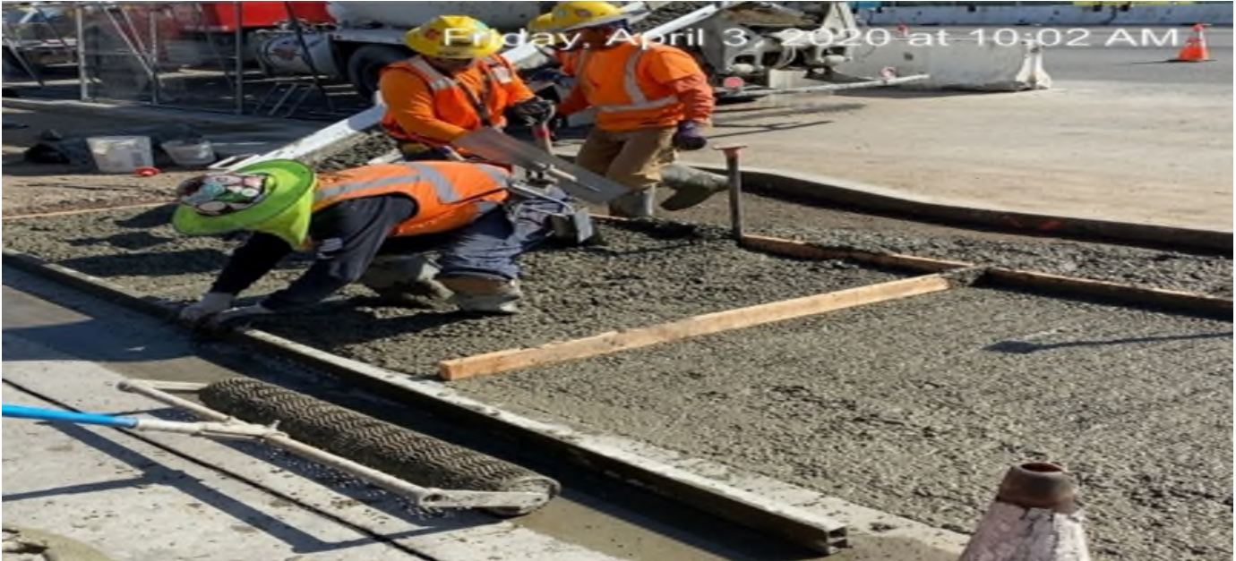
EXPO STATION – Placing concrete for new curb/gutter and driveway installation on southbound Crenshaw Blvd between Exposition Blvd and Rodeo Blvd.
