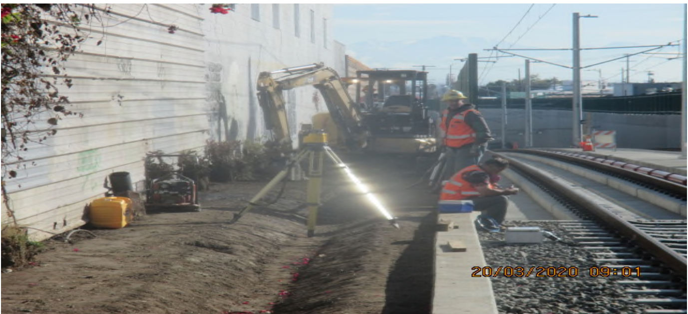
UG3 – Excavating for culvert drainage along the bottom of the southbound barrier wall in preparation for concrete placement. 3/20/20
