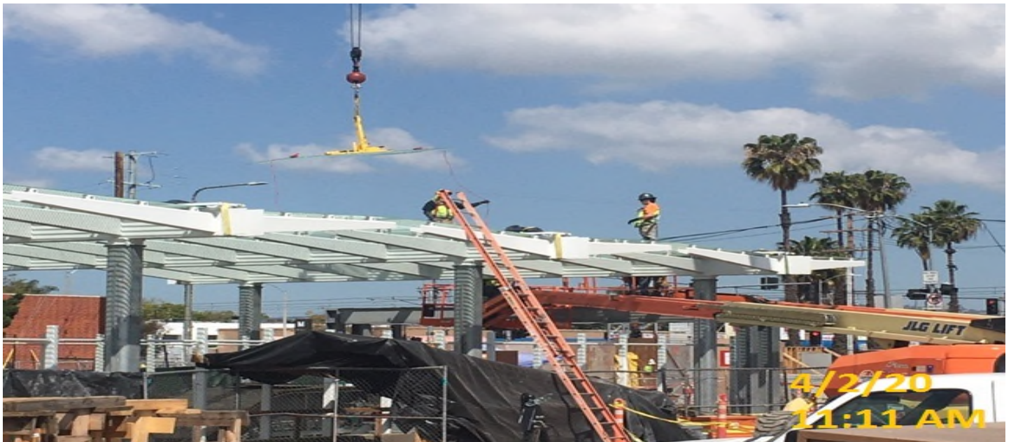
EXPO STATION – Continue tempered glass installation on top of the main entrance canopy at the plaza level.
