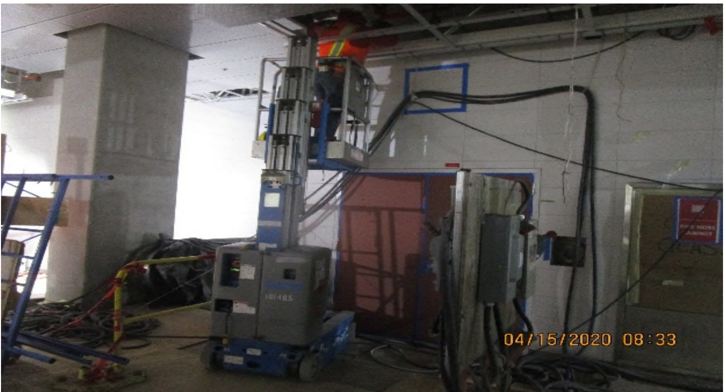
Crenshaw/MLK - MLK, Concourse Paid Area C146, resume rough in 3/4" flex whips to Williams light cover fixtures at drop ceiling.
