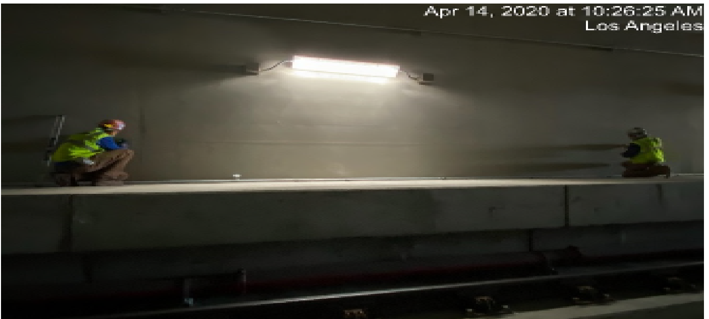
UG4 – Began layout for handrail installation for the emergency walkways along the southbound tunnel.
