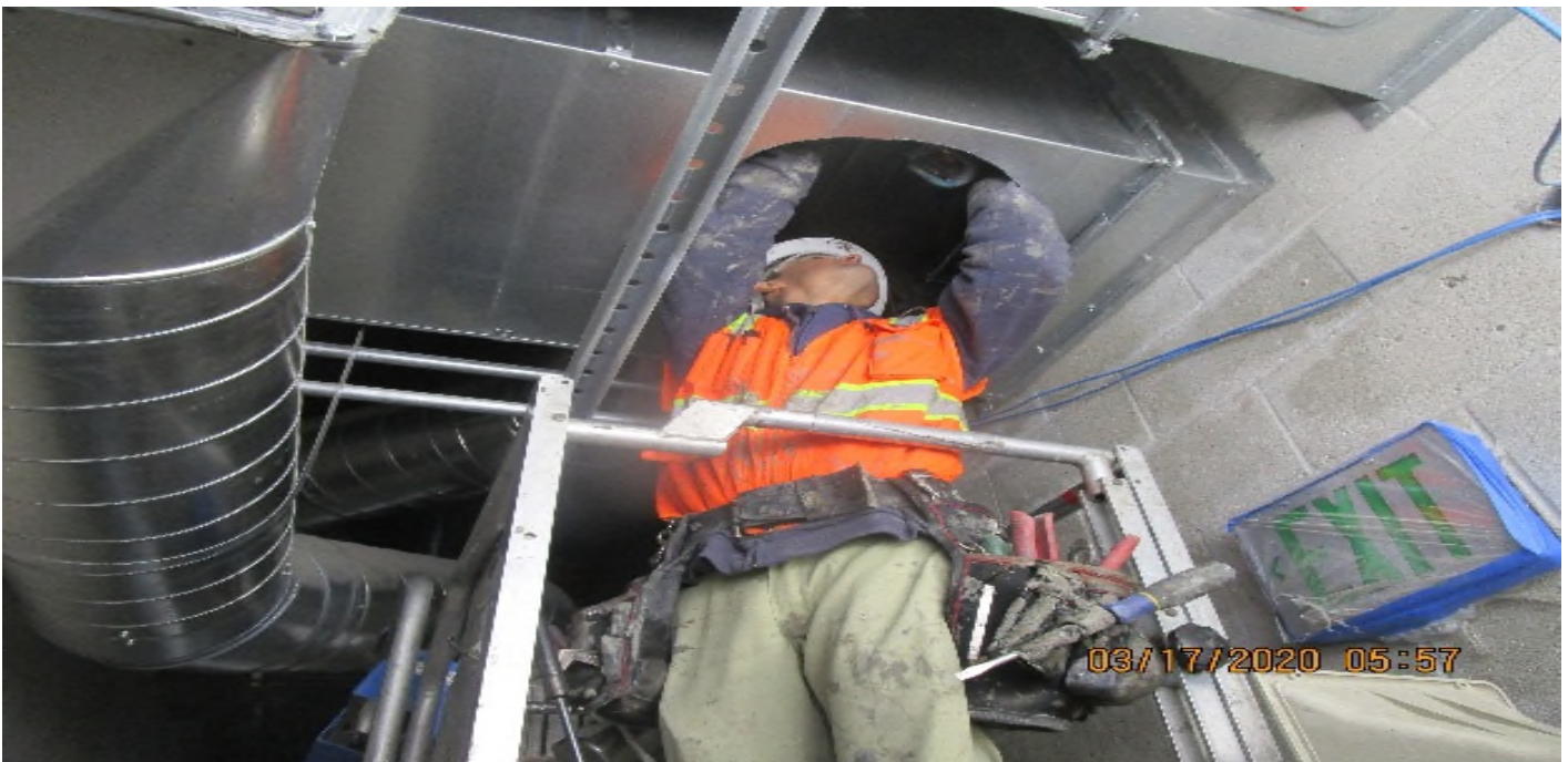
Crenshaw/Vernon - Vestibule #2 C108, begin cut in 24"x24" oval EA access doors (upper & lower) for F.A JB access.
