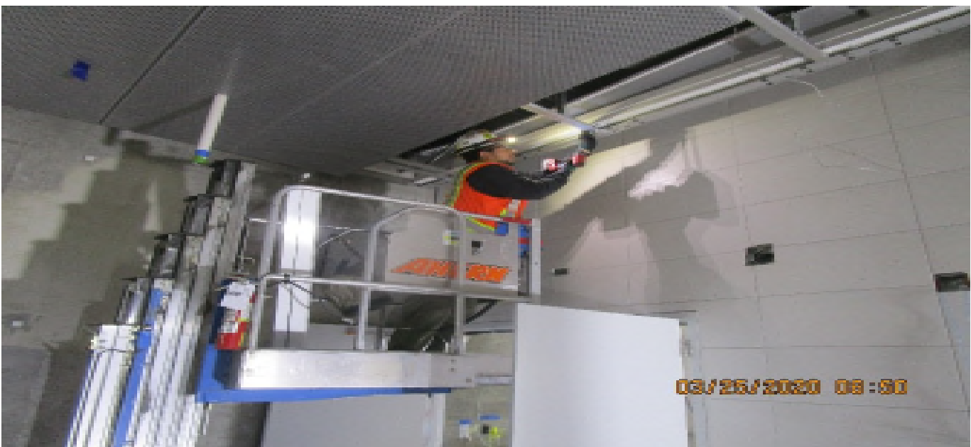
MLK STATION – Continue installing light cove and ceiling panels throughout the Free & Paid Area of the concourse level.
