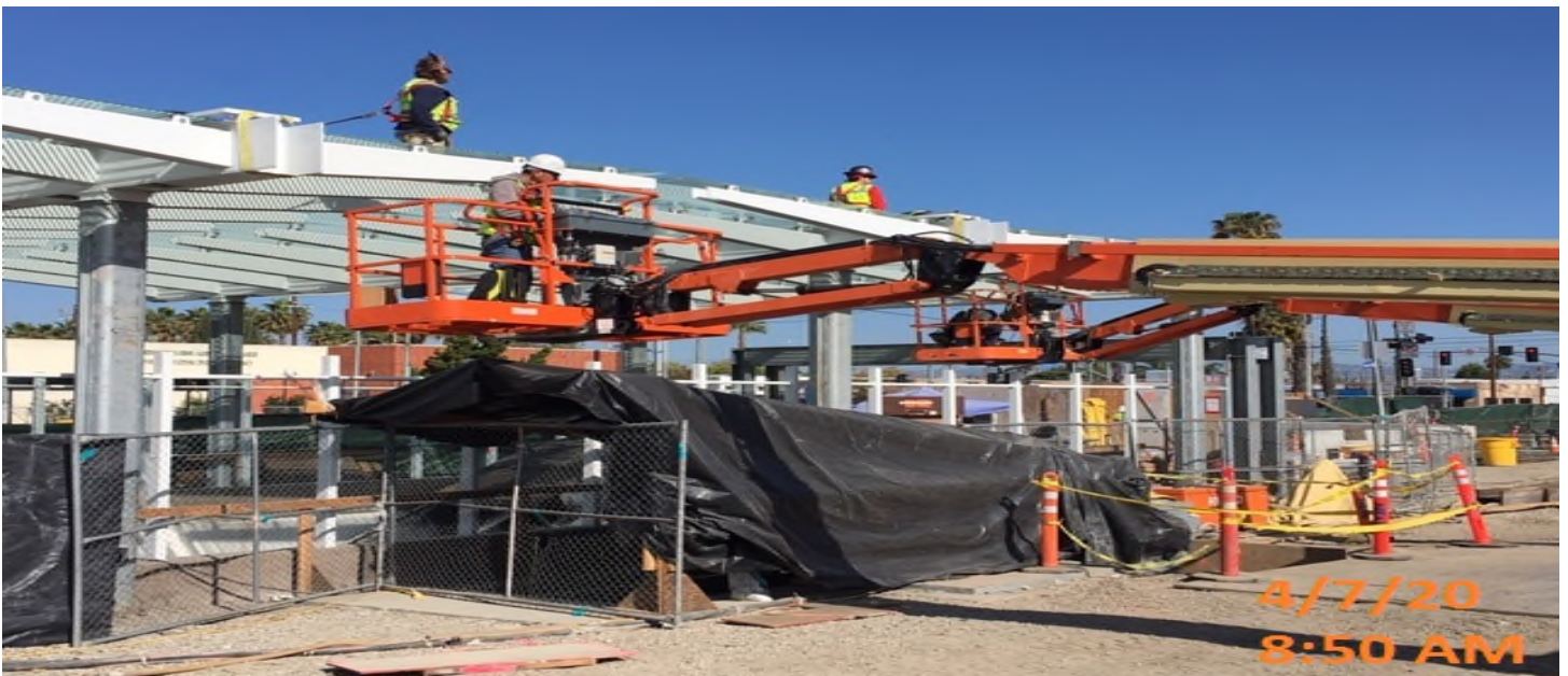
EXPO STATION – Caulking glass panel edges with silicone on top of the main entrance canopy at the plaza level.
