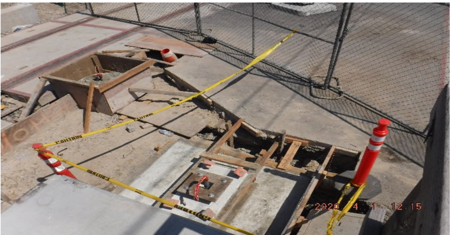
Florence/West – STA 267+40 right shoulder TK#3-SB looking north – track sub-structure disturbance around newly build pole foundation PUNCH LIST
