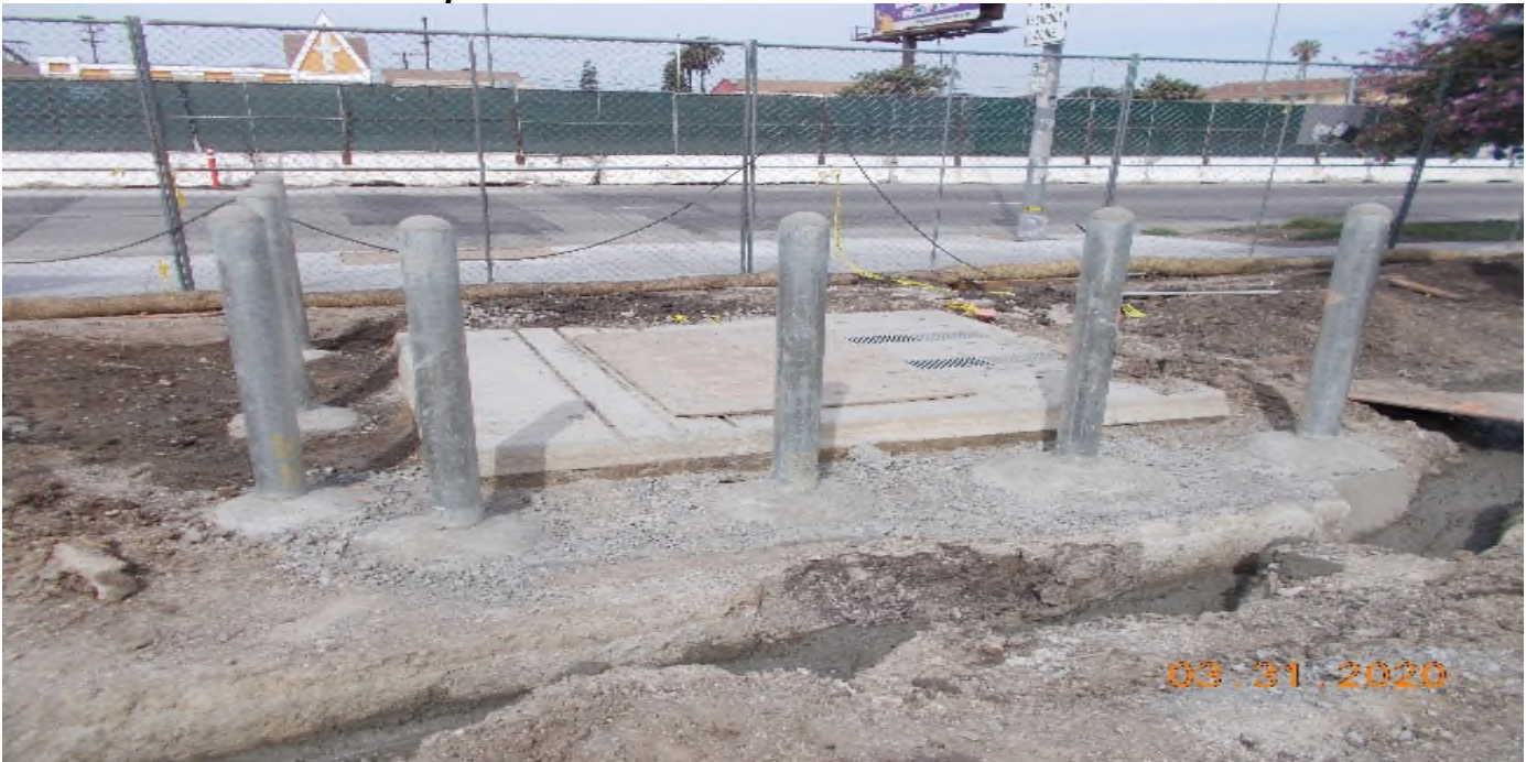
PARK MESA – Completed bollard installation around the DWP transformer pad at TPSS#7 on 60th St & Crenshaw Blvd.
