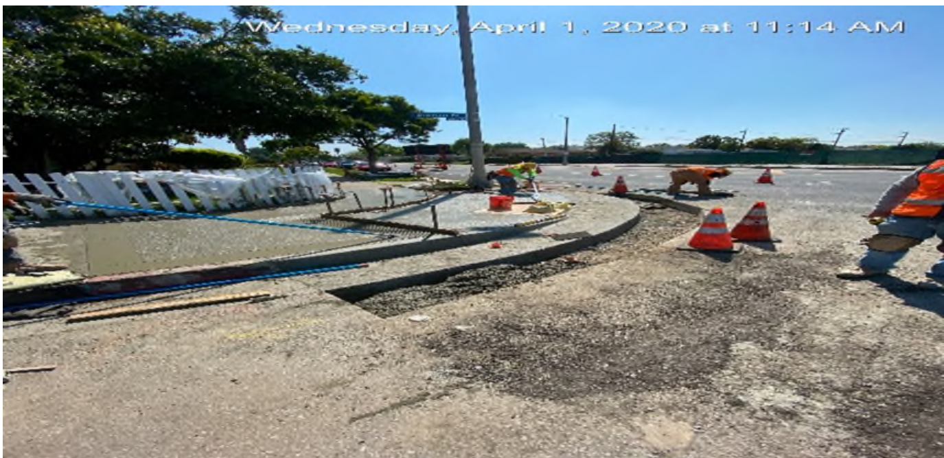
EXPO STATION – Continue concrete placement for new curb/gutter and ADA ramp installation on Bronson Ave east of the plaza.
