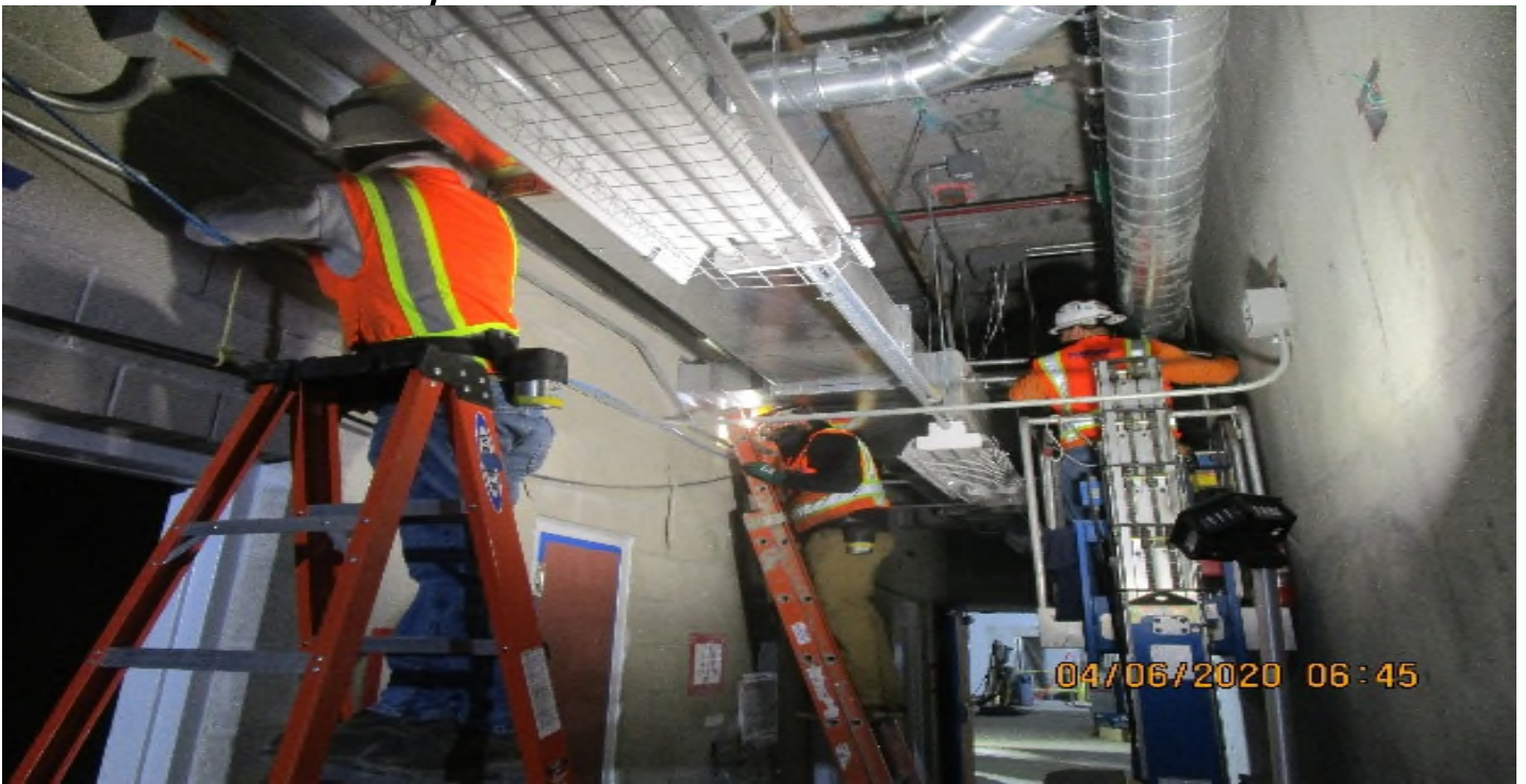
Crenshaw/MLK - Corridor C120, Rough in anchors, supports & Pipping 1" GRC to device locations for fire alarm strobes.
