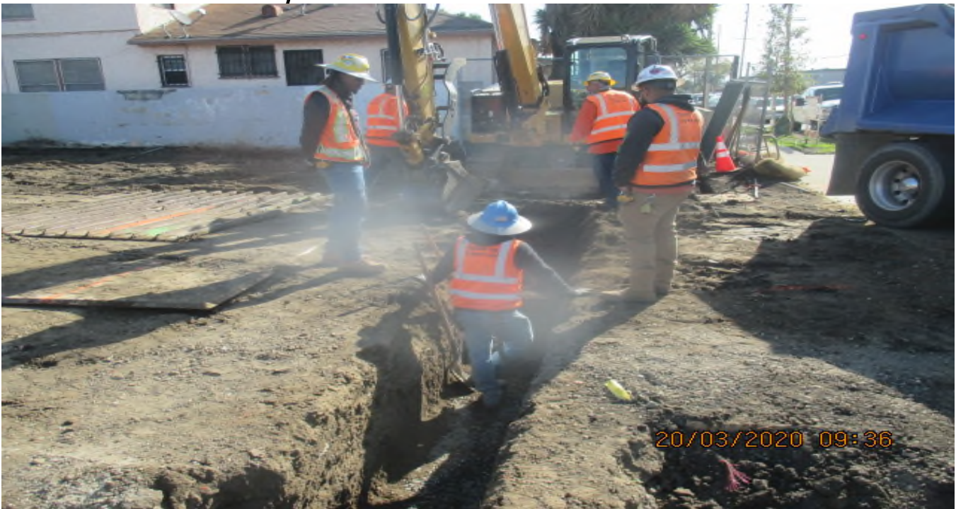
PARK MESA – Continue excavating for the 12” HDPE storm drain line N-12 at TPSS#7 on 60th St & Crenshaw Blvd. 3/20/20
