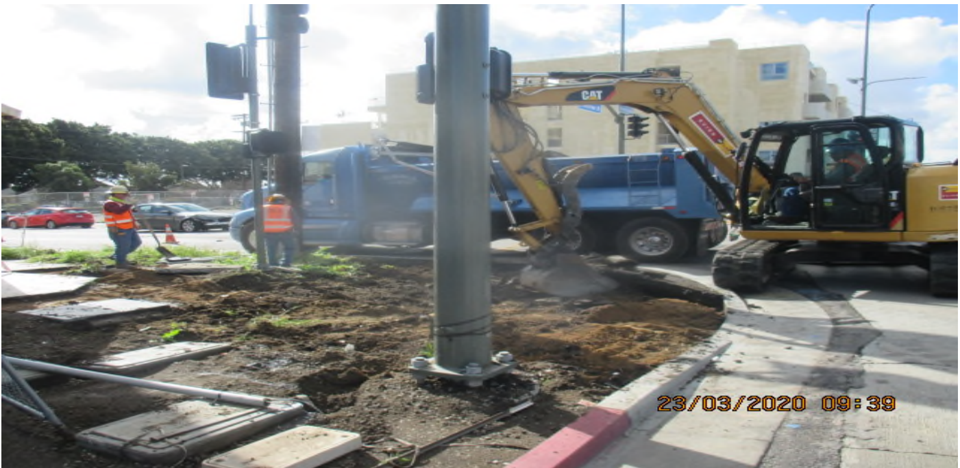
PARK MESA – Excavating for new sidewalk and ADA ramp installation on the northeast corner of 54th St and Crenshaw Blvd. 3/23/20
