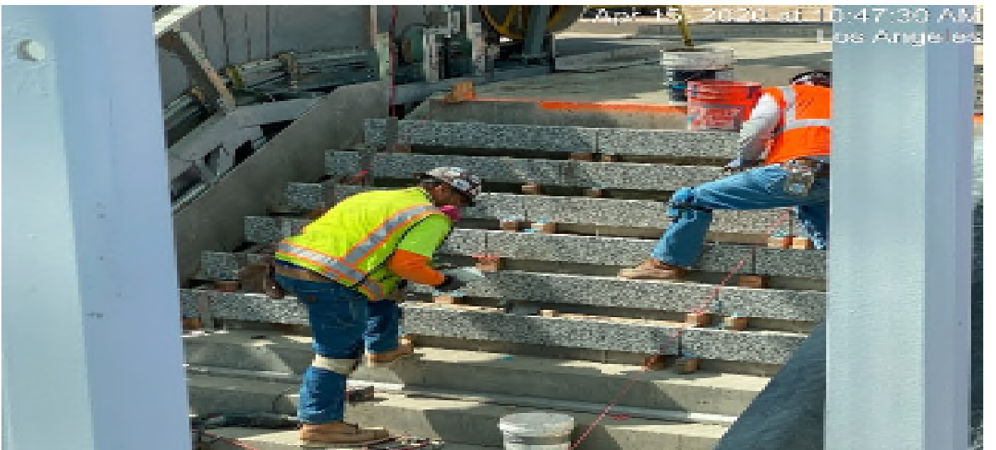
LEIMERT PARK STATION – Continue granite thread and riser installation at the main stair case landing of the plaza level.
