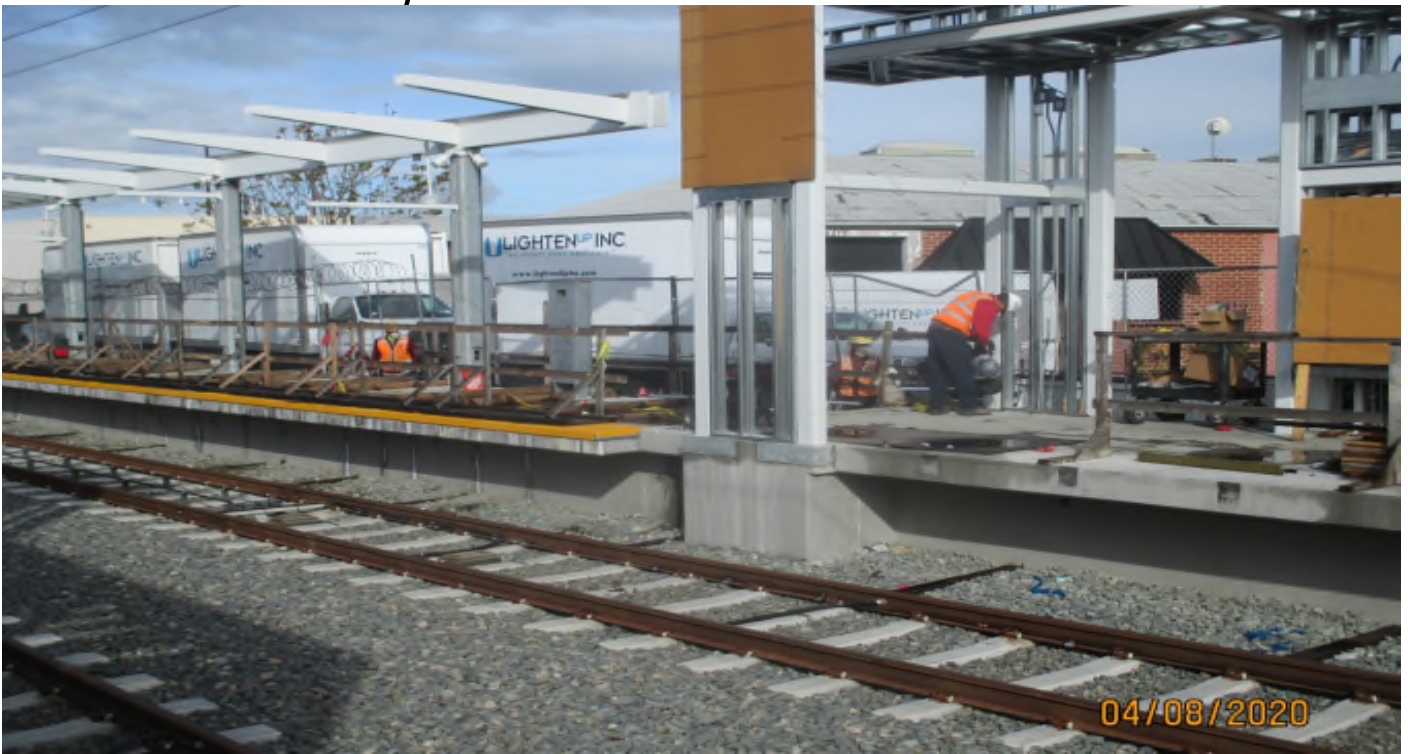
Florence/Hindry – Fence post anchor removal at the SB platform of the Hindry Station.
