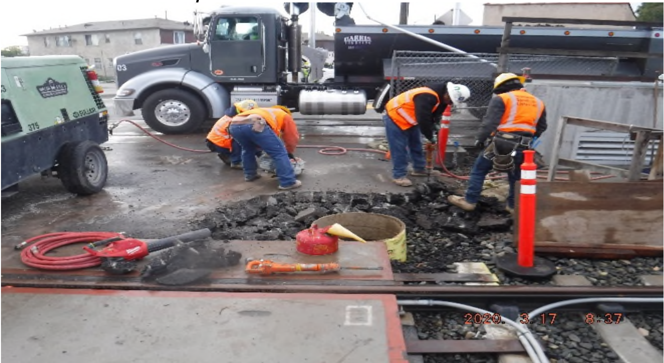
Florence/West – Select Electric Place conc foundation for controller at Redondo and West
