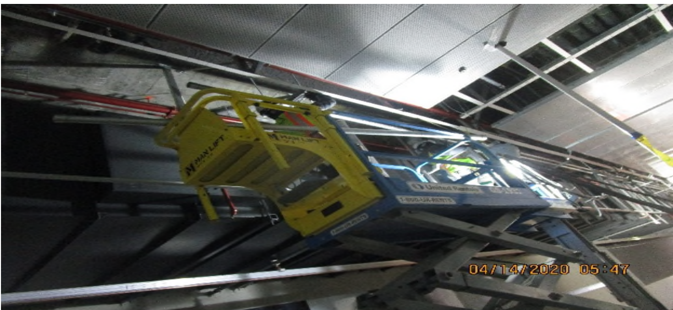
LEIMERT PARK STATION – Continue radiax cable conduit and support rack installation on the platform ceiling level.
