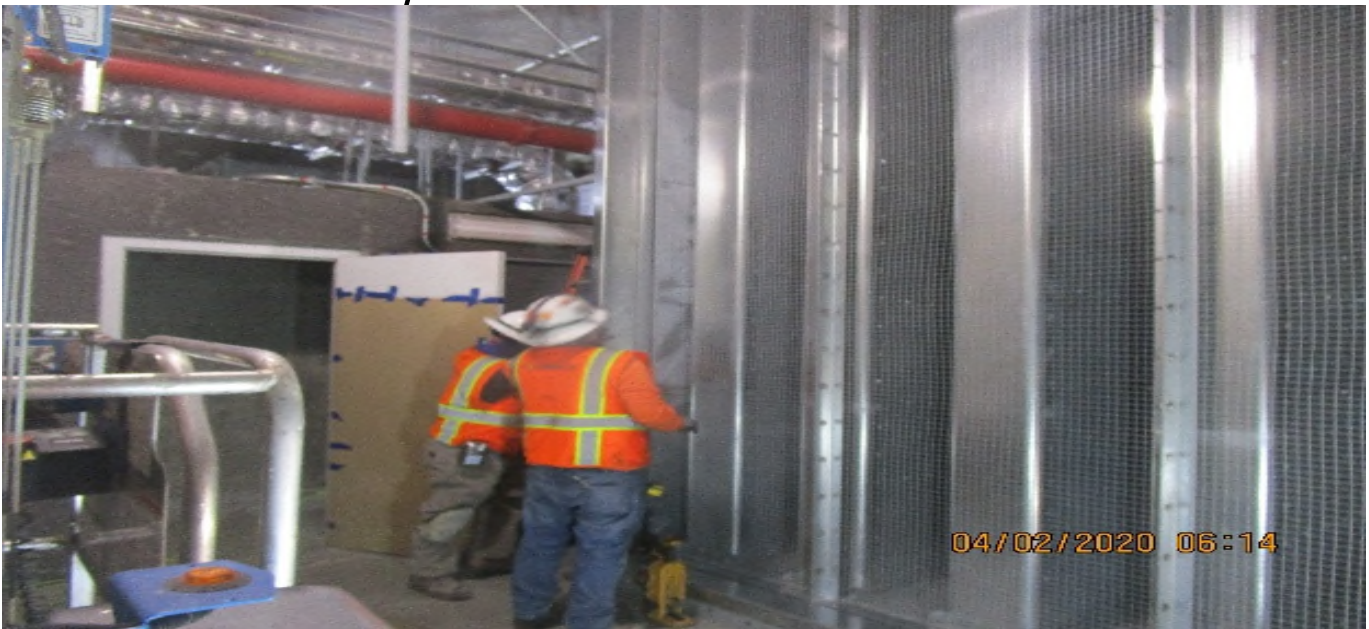
LEIMERT PARK STATION – Continue installing bird screen protection to the sound attenuator for EVF-6-301 in the South Fan Room C – 102 of the concourse level.
