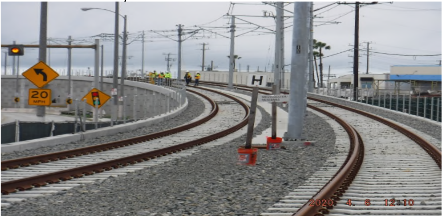
Manchester Bridge – STA 131+00 TK#4-NB looking south - checking rail grinding profile north ramp Manchester Bridge.
