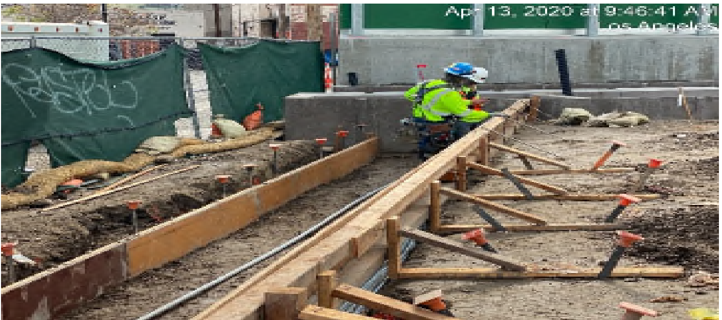
LEIMERT PARK STATION – Continue formwork for the planter section stair risers at the plaza level.
