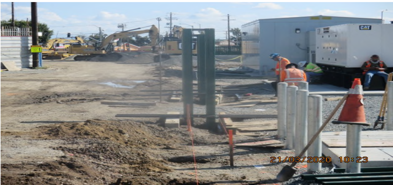
UG3 – Installing fence posts around the Auxiliary power site perimeter adjacent to the south end portal entrance. 3/21/20
