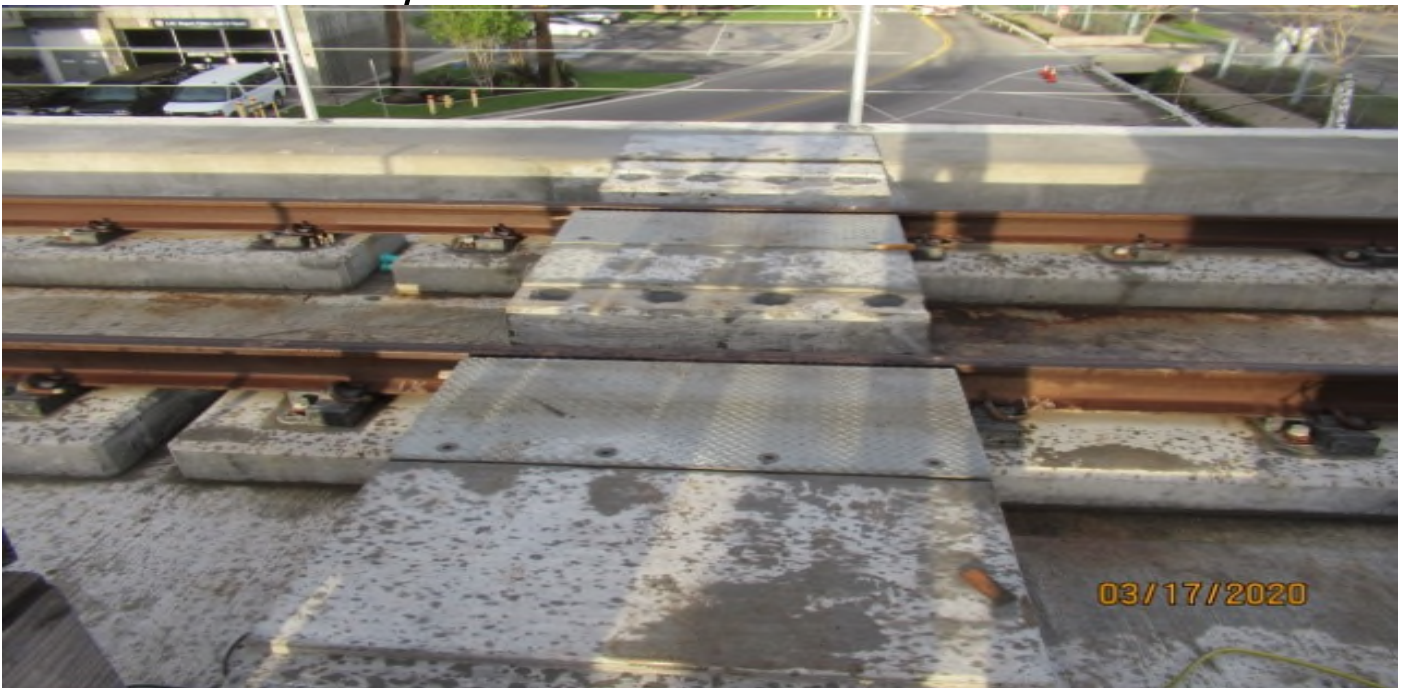
Aviation/Century – SB #3 track STA 66+19 Century-Aviation bridge, incomplete install of Ped. Crossing plates & inserts (looking west).
