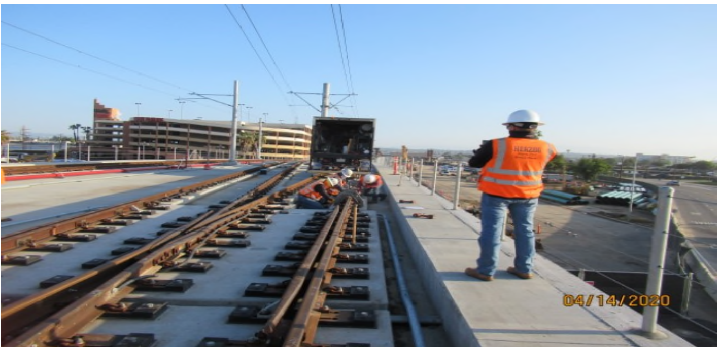
Aviation/Century – HCC, repairing cross levels on 10K1LH XO Century-Aviation Bridge NB # 4 track.
