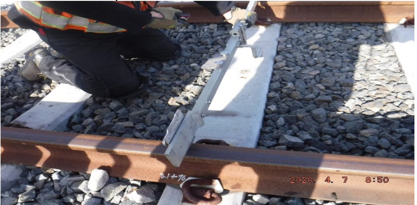
Aviation/Century – STA 21+96 TK#4-NB looking west – checking rail grinding CPC on tangent -Aviation
