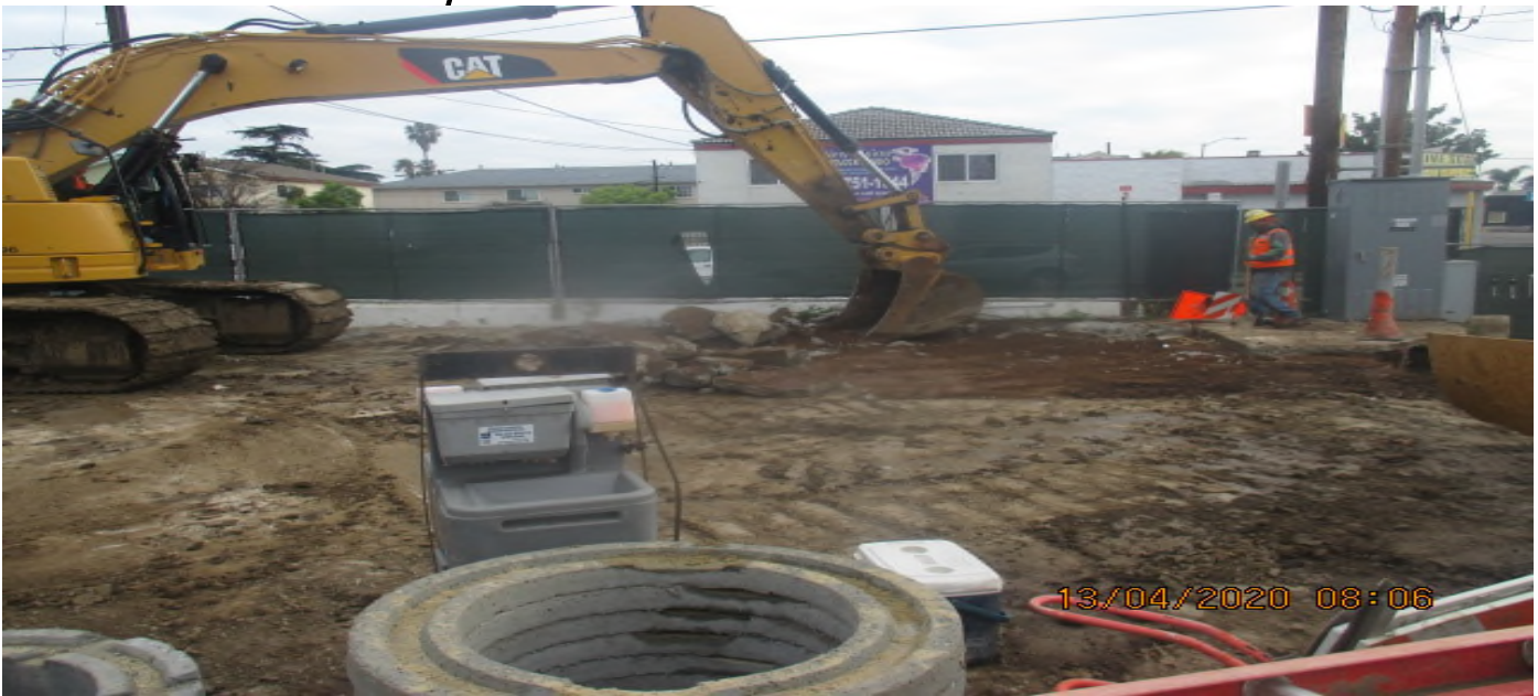
UG3 – Continue grading and excavating for the culvert drainage along the eastbound sidewalk of 67th St in preparation for concrete placement. 4/13/20
