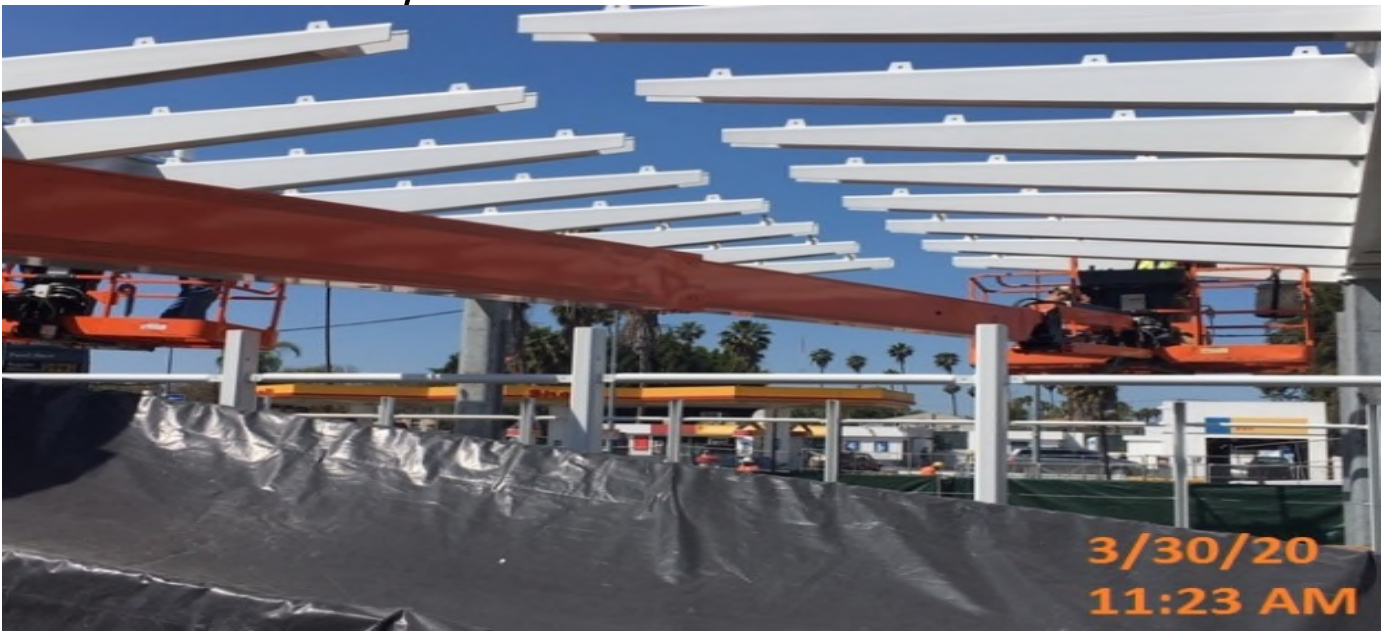
EXPO STATION – Installing glass panel fittings for the main entrance canopy at the plaza level.
