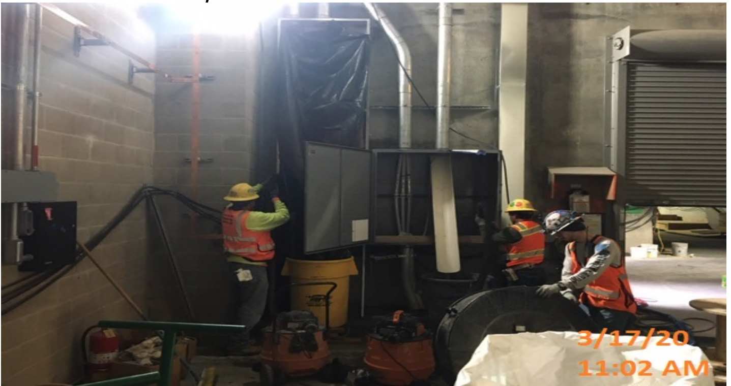
Crenshaw/Expo - WSCC crew doing exploratory work on water intrusion into TPSS room.
