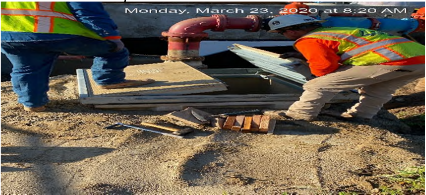
MLK STATION – Installing concrete thrust block supports on top of the fire protection vault at the plaza level.
