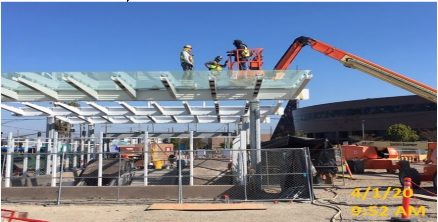
EXPO STATION – Began tempered glass installation for the main entrance canopy at the plaza level.
