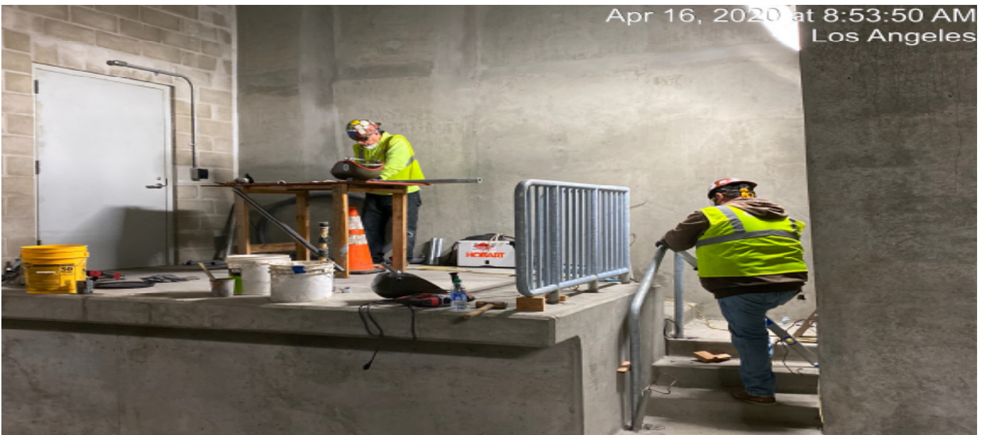
UG3 – Continue installing handrails for the Sump Pump Rooms for both north and southbound tunnels.
