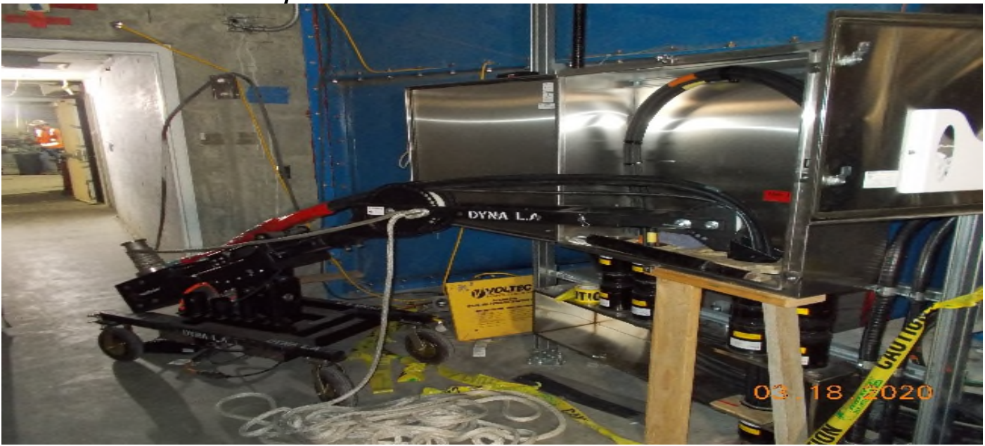
EXPO STATION – Continue installing fire rated conduit to the pull box for the EVFs in the North Fan Room C – 102 of the concourse level.
