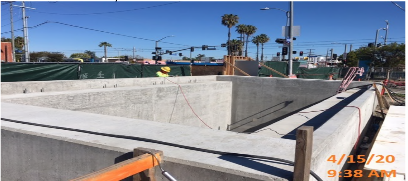
EXPO STATION – Surfacing walls of the north emergency ventilation shaft at the plaza level.
