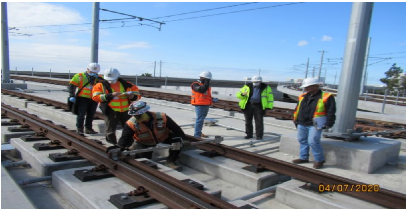
Guideway - Site walk for field verification of rail profile radius on NB1300 track STA 12+56 at GL Wye
