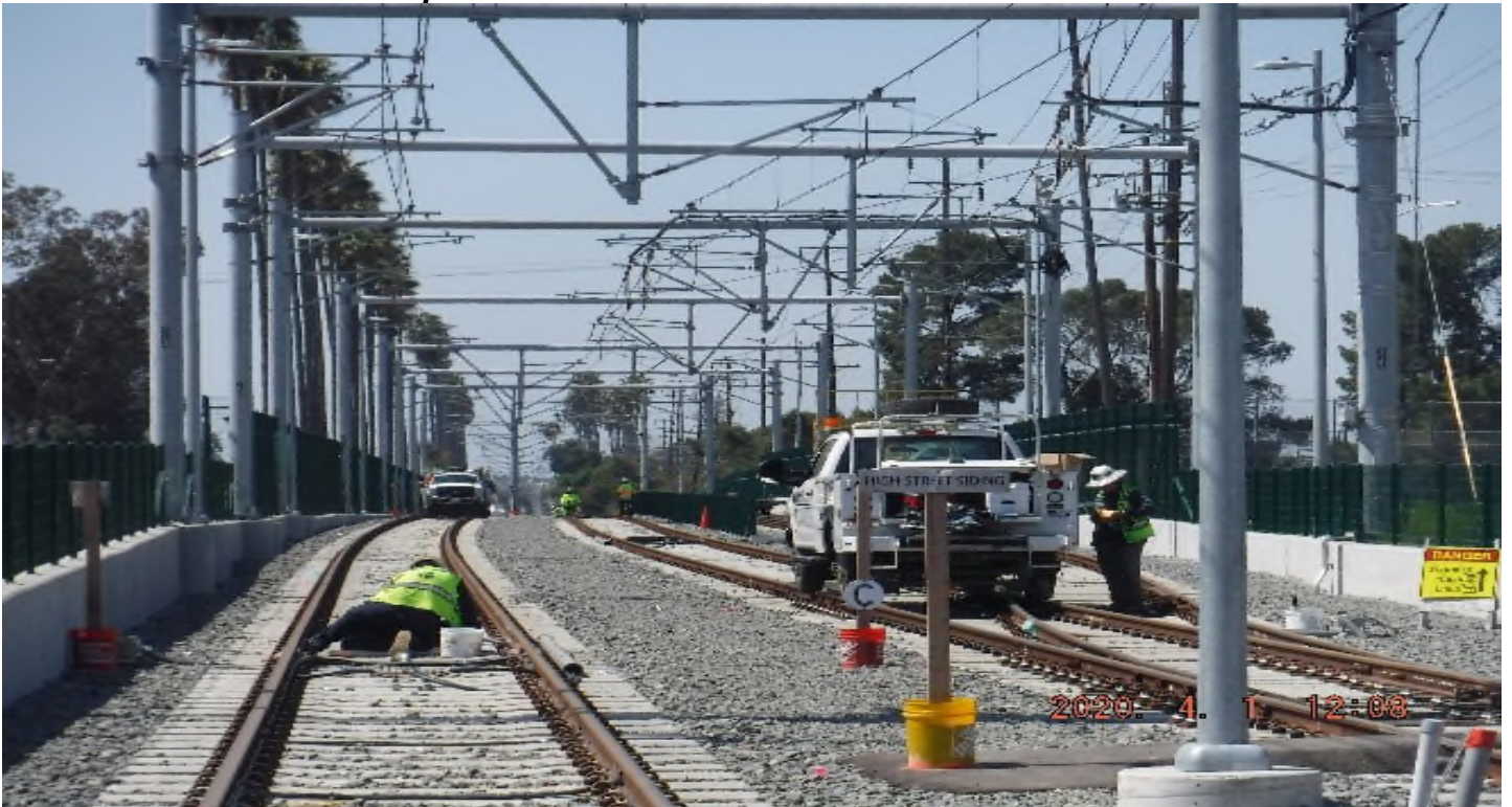
Florence/High St. - STA 256+20 TK#4-NB looking south – system work south of High St at grade crossing - Siding Track.
