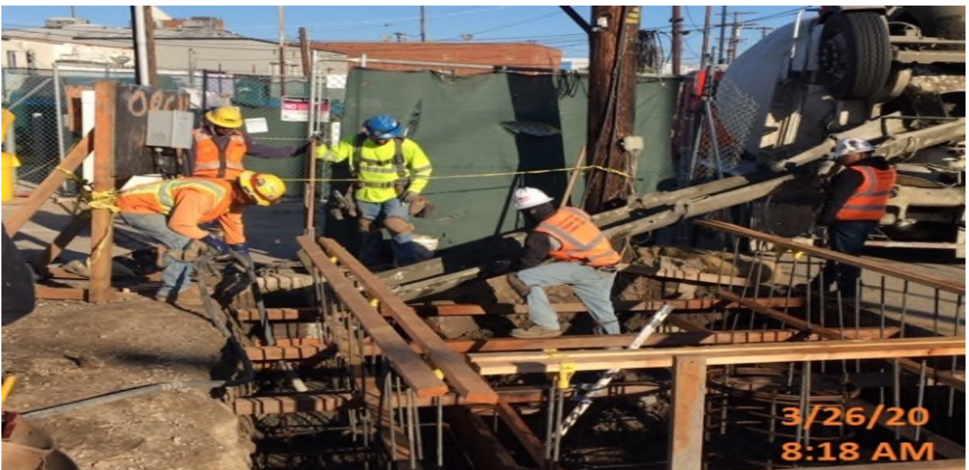
LEIMERT PARK STATION – Placing concrete for the planar wall and footings at the east side of the plaza level.
