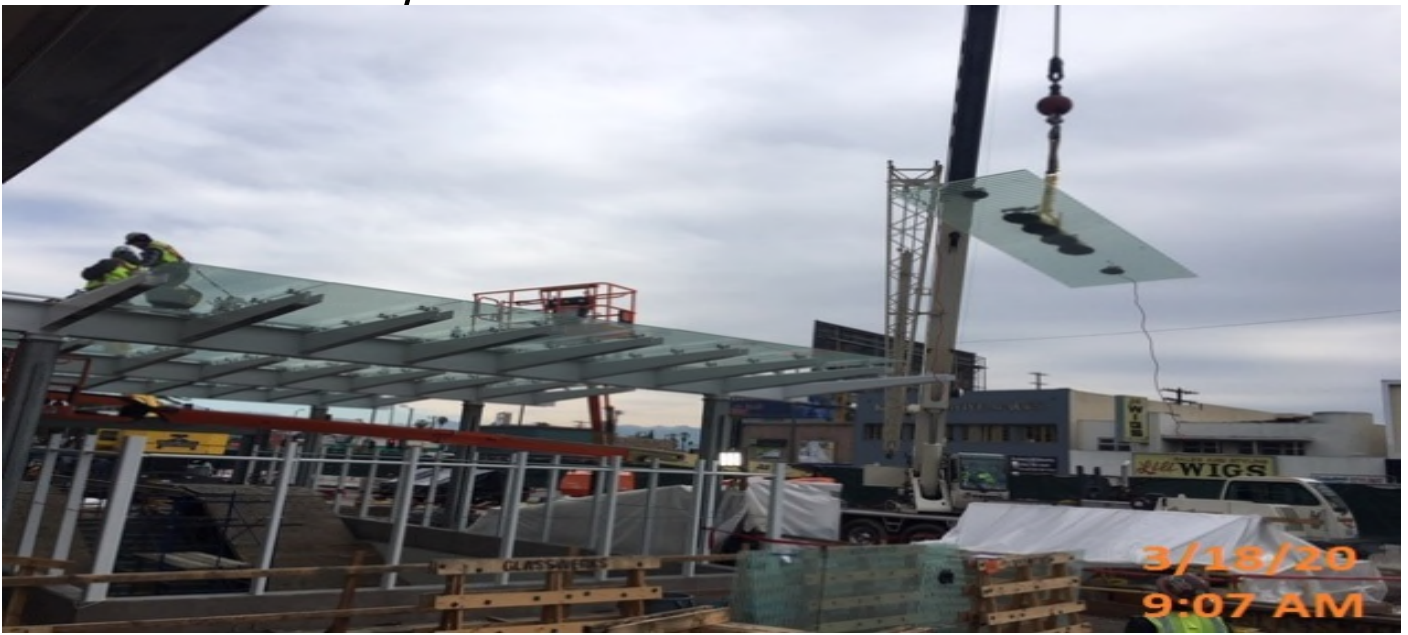
MLK STATION – Began tempered glass installation above the main entrance canopy structure at the plaza level.
