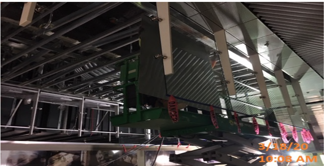
LEIMERT PARK STATION – Continue installing stainless steel cladding panels on the platform ceiling level.
