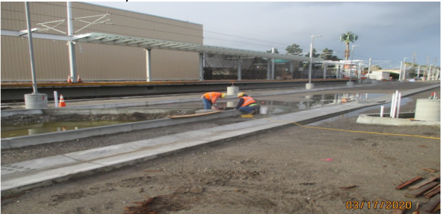
Florence/West – Chipping away the encased electrical conduit at the West Station. Facing SW.
