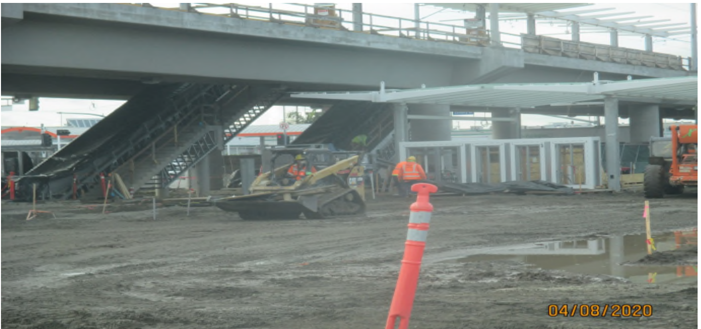
Aviation/Century – SWPPP operations and prep for the rain at the Aviation station yard.
