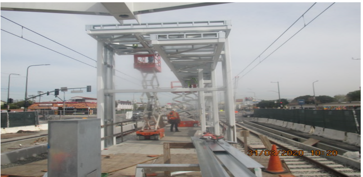
Hyde Park Station – Installing light gauge framing and roofing on the north end canopy structure. 3/30/20
