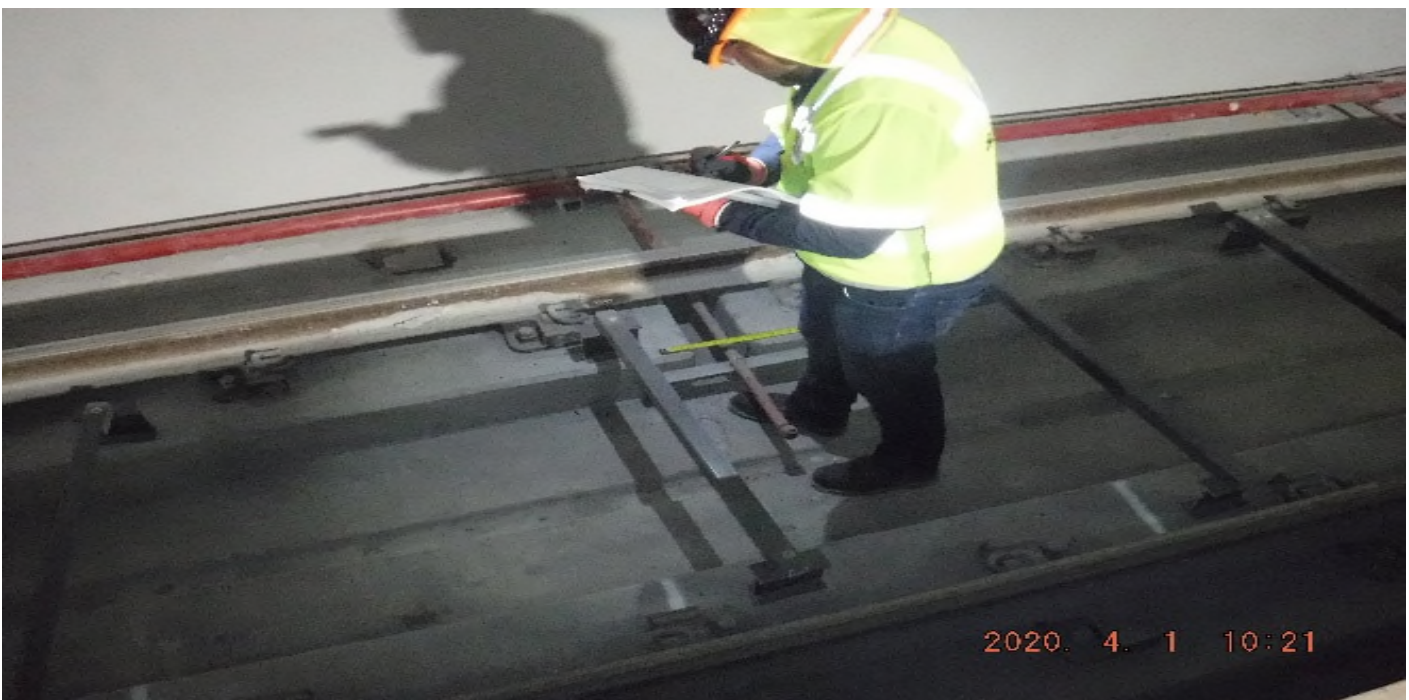
Crenshaw/Expo - STA 447+80 TK#4-NB looking east – record data after plinth rebar scanning UG4 Exposition Station.
