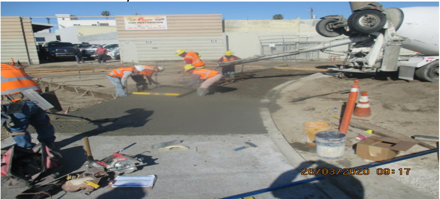
UG3 – Installed block-out forms and place concrete for new Victoria Cul-de-sac sidewalk and driveway installation. 3/26/20
