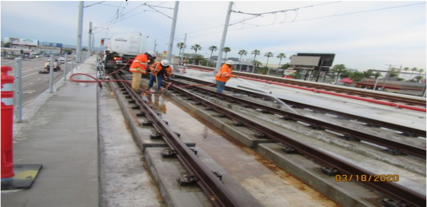
Aviation/Century – HCC using hi-rail water truck to remove excess debris from guideway on Century-Aviation deck thru 10K1LH XO (looking southwest)
