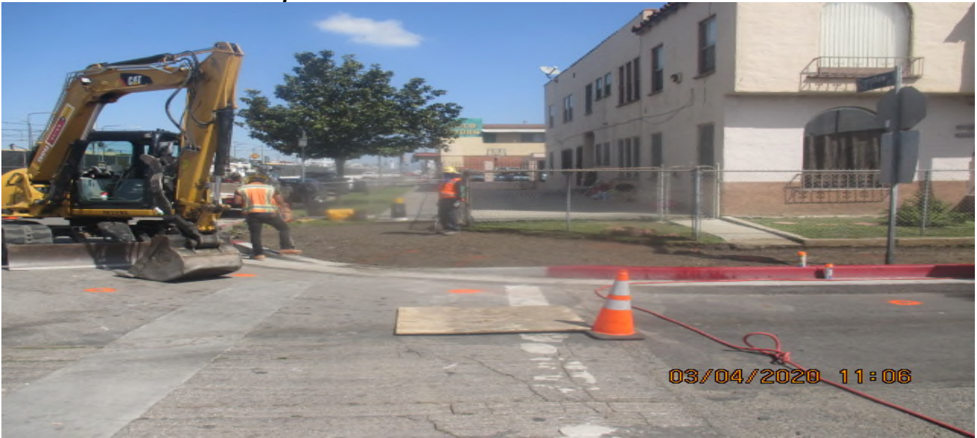
PARK MESA – Excavating/grading in preparation for concrete placement for new sidewalk and ADA ramp installation on the northeast corner of 59th Pl & Crenshaw Blvd. 4/3/20
