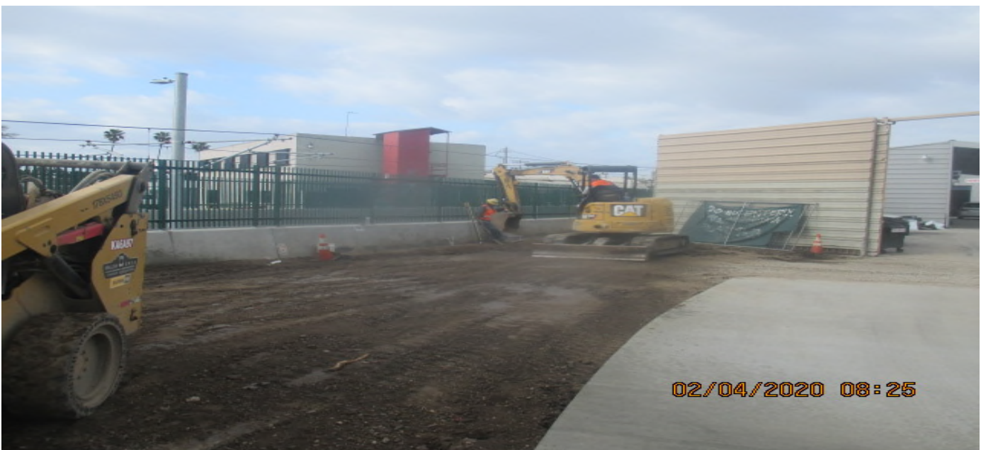
UG3 – Continue grading and excavating for the culvert drainage along the southbound barrier wall in preparation for concrete placement. 4/2/20
