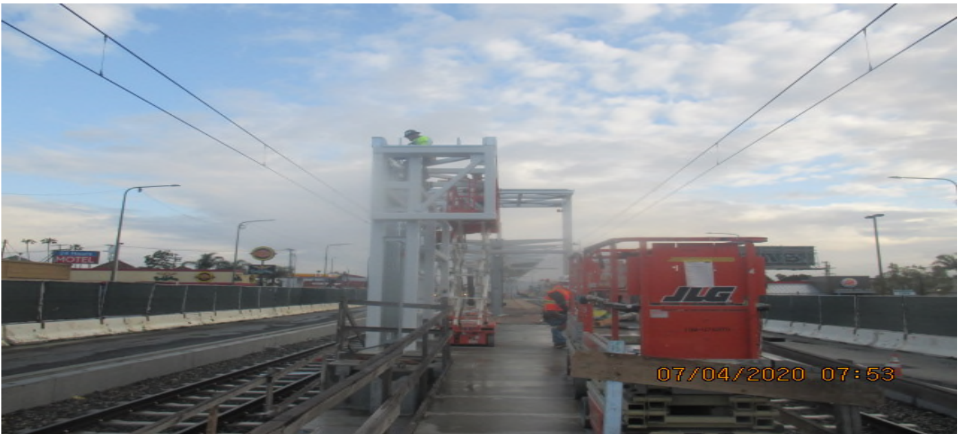
Hyde Park Station – Continue installing light gauge framing and roofing on the south end canopy structure. 4/7/20
