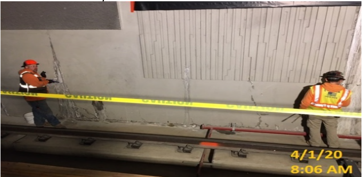
Crenshaw/MLK - Hayward Baker removing polyurethane crack-cold joint grout injections packers at platform level.
