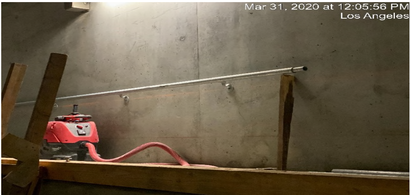
UG3 – Continue installing and welding handrails for the emergency walkway at the northbound tunnel at Sta 300+50.
