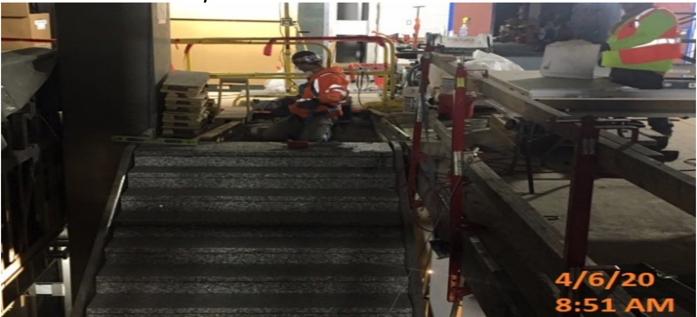
MLK STATION – Installing granite treads and landing sections to staircase #3 at the concourse level.
