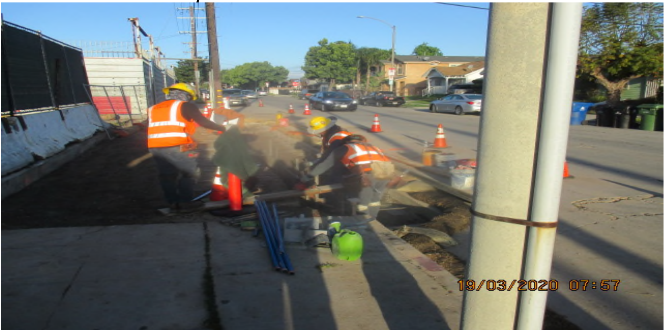
UG3 – Continue new sidewalk/driveway installation on the southwest corner of 67th St and Crenshaw Blvd. 3/19/20
