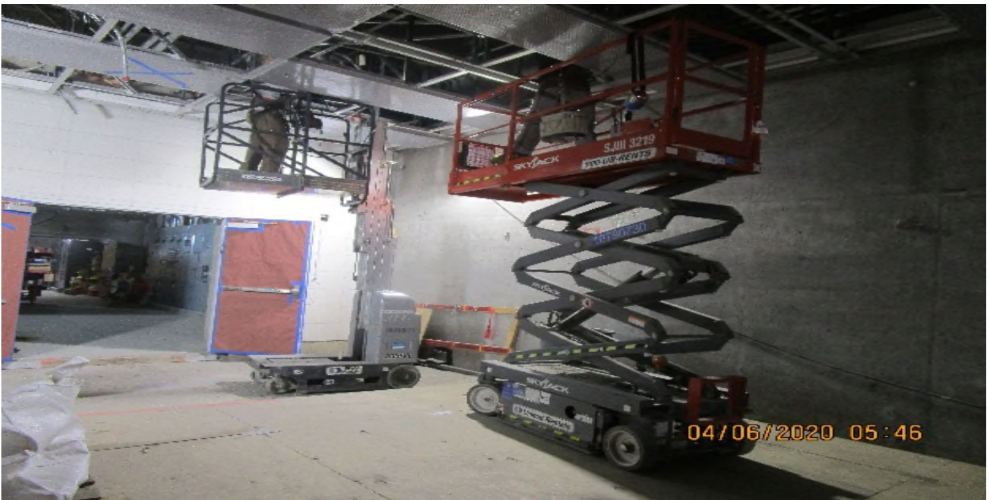
Crenshaw/MLK - MLK Concourse, Paid Area C119 continued rough in Radiax & coaxial cable conduit support racks.
