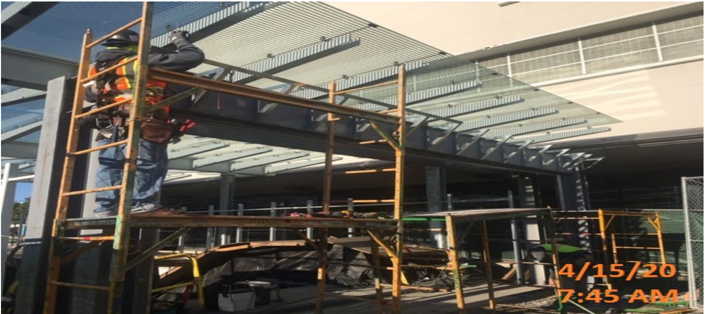
MLK STATION – Continue installing the overhead ceiling grille to the main entrance canopy at the plaza level.
