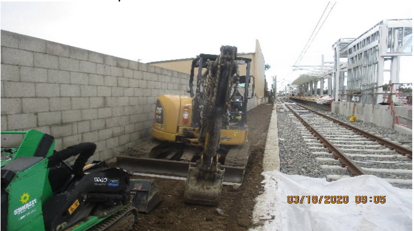
Florence/West – WSCC Make grade for swale at outside of Balast wall at West Sta
