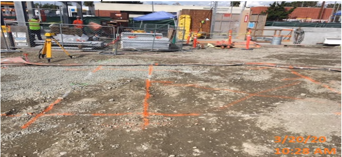
EXPO STATION – Setting grid lines in preparation for underground electrical vault and fiber installation for duct banks M02 & M07 at the plaza.
