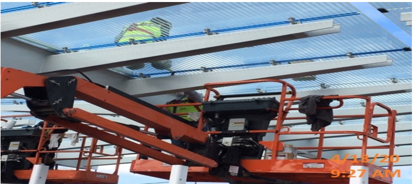
EXPO STATION – Continue caulking glass panel edges with silicone on top of the main entrance canopy at the plaza level.
