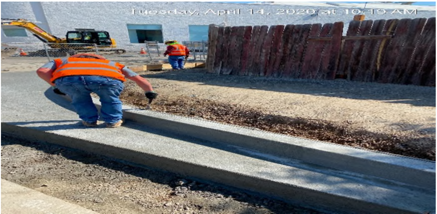
EXPO STATION – Fine grading soil for the new sidewalk and ADA ramp installation on Bronson Ave east of the plaza.
