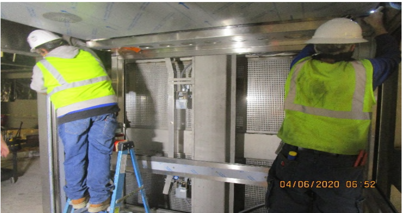
Crenshaw/MLK - MLK Platform, Elevator 3 & 4, continued install cab car canopy panel sections & car operating control panel.
