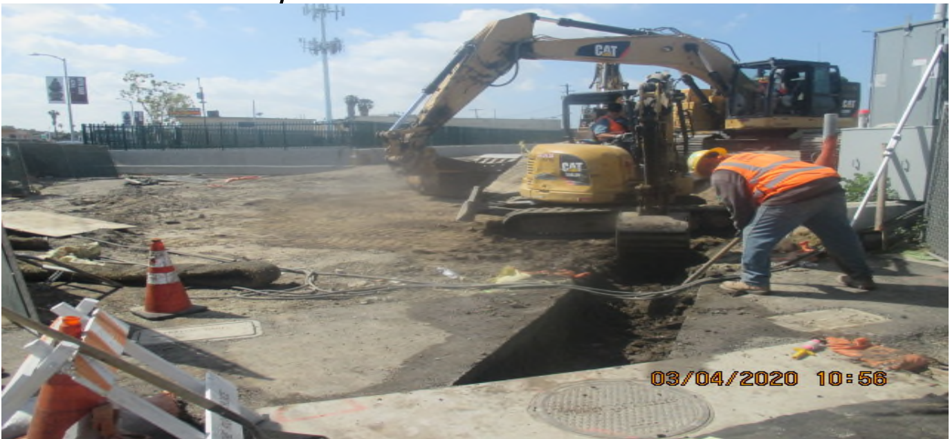
UG3 – Excavating for 18” HDPE drain line connection to Catch Basin #1 on the southwest corner of 67th St and Crenshaw Blvd. 4/3/20
