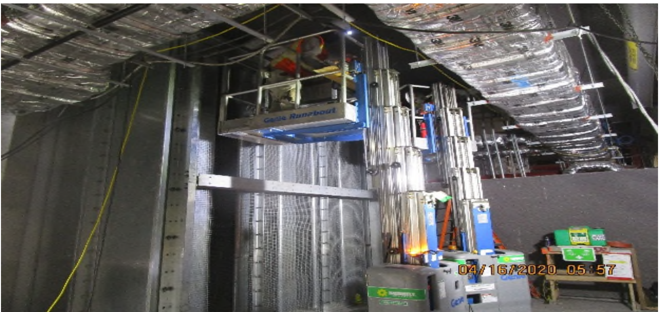
LEIMERT PARK STATION – Began rough-in of support framing and hardware for the tunnel fan dampers in the South Tunnel vent Plenum C – 104 of the concourse level.
