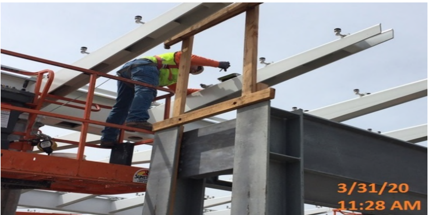
EXPO STATION – Continue installing glass panel fittings for the main entrance canopy at the plaza level.
