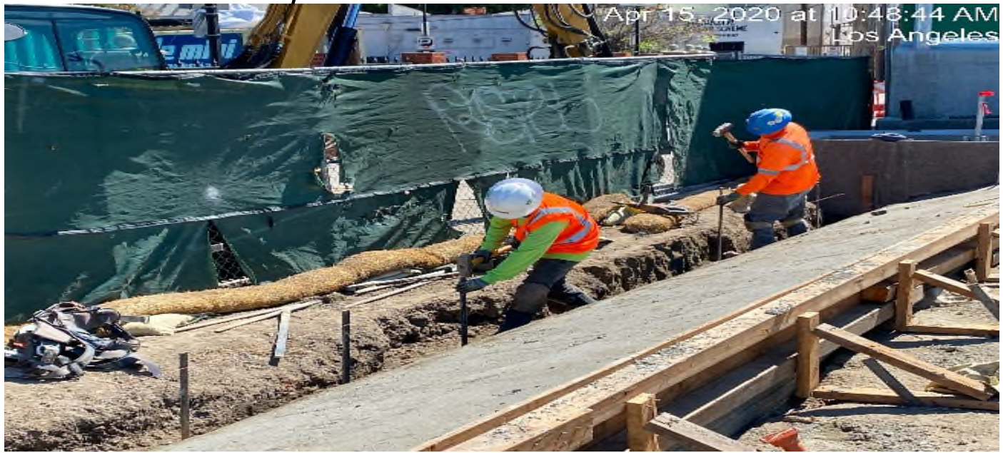
LEIMERT PARK STATION – Continue formwork for the planter section stair risers at the plaza level.
