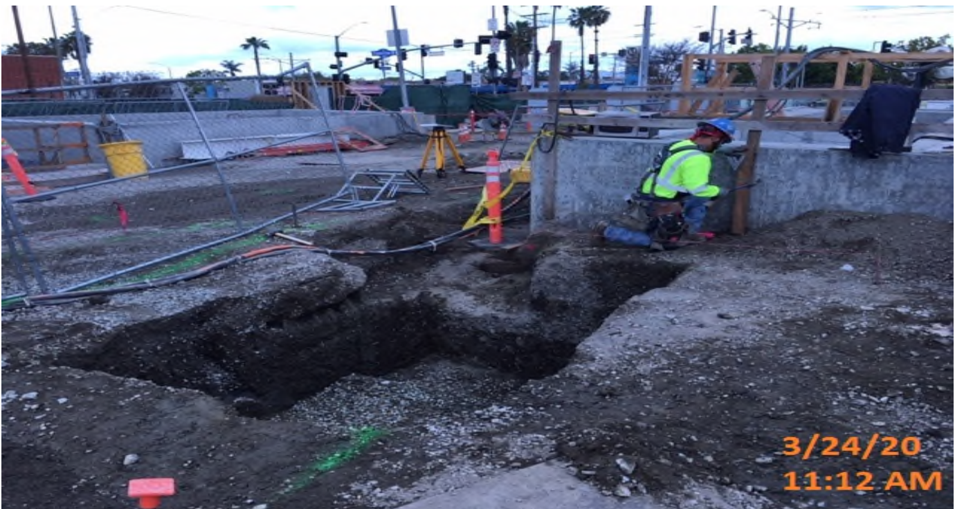
EXPO STATION – Continue trenching in preparation for underground electrical vault and fiber installation for duct banks M02 & M07 at the plaza.
