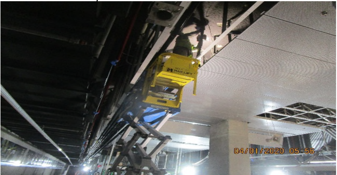
Crenshaw/Vernon - Vernon Platform, northbound, north platform continued rough in Radiax & coaxial cable conduit support racks
