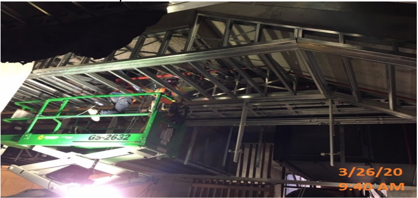
EXPO STATION – Continue installing stainless steel cladding panels on the platform ceiling level.
