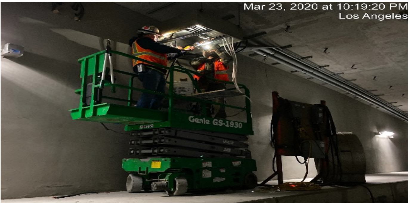
UG-4- Continue splicing wires for the tunnel booster junction boxes at the southbound tunnel at Sta 374+00.
