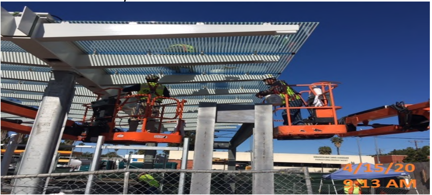
EXPO STATION – Finalizing glass panel caulking on top of the main entrance canopy at the plaza level.
