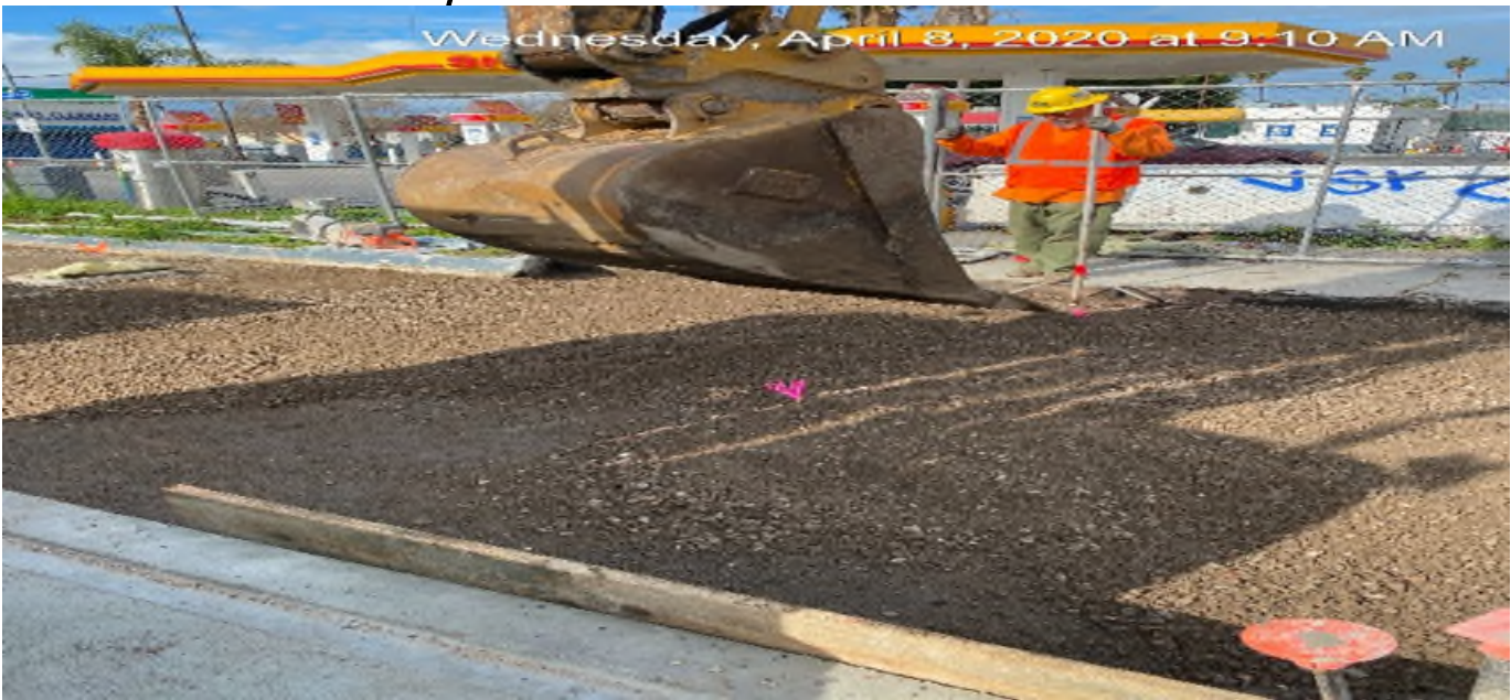
EXPO STATION – Backfilling and grading/compacting driveway on southbound Crenshaw Blvd between Exposition Blvd and Rodeo Blvd.
