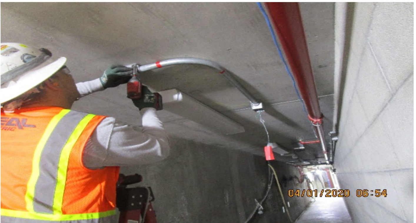
Crenshaw/MLK - MLK Concourse, Corridor 1080 Continued pipping 1" GRC & rough in 4S malleable steel JBs for smoke & strobes.
