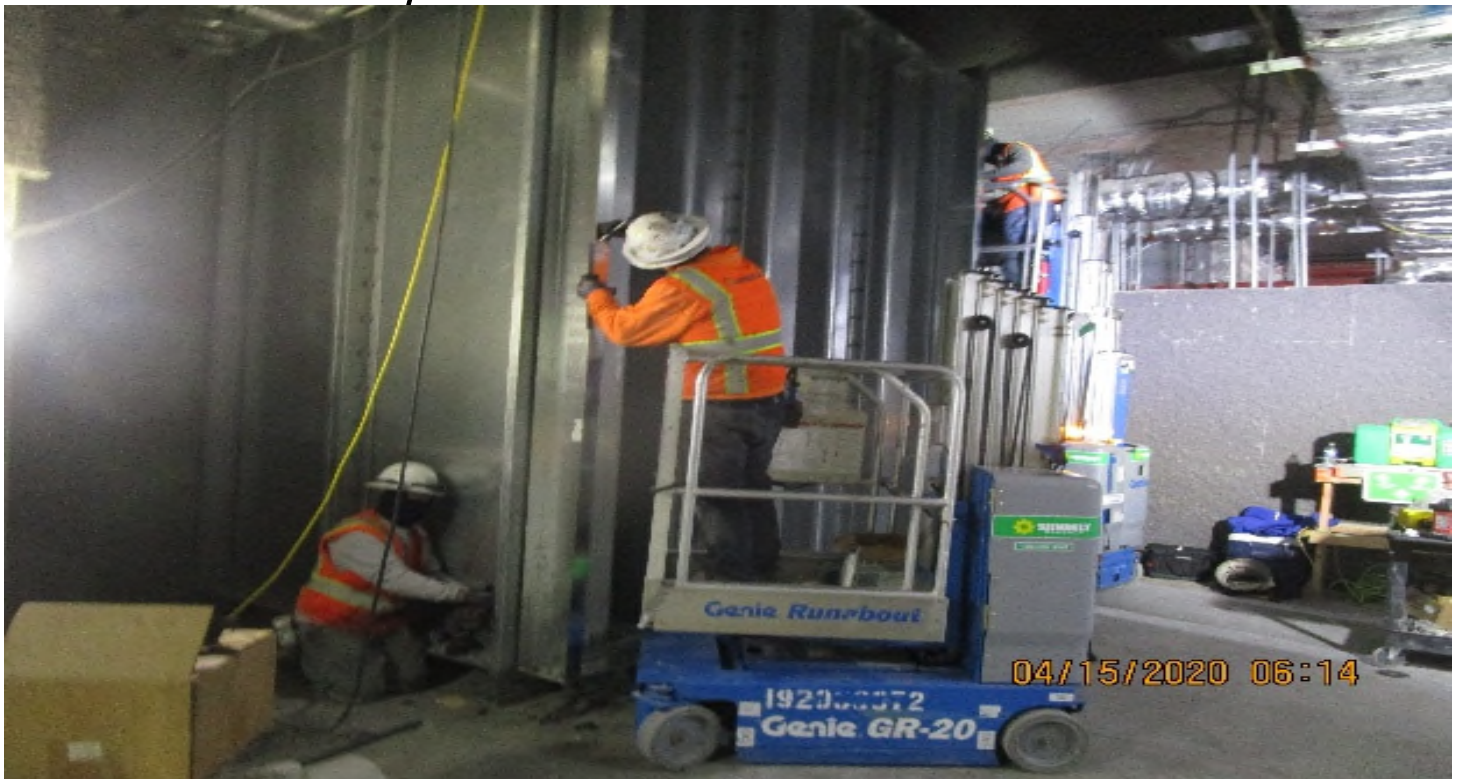
Crenshaw/Vernon - Concourse, Tunnel vent plenum (S) #2 C106, TFD-6-101 begin rough in framing & support hardware.
