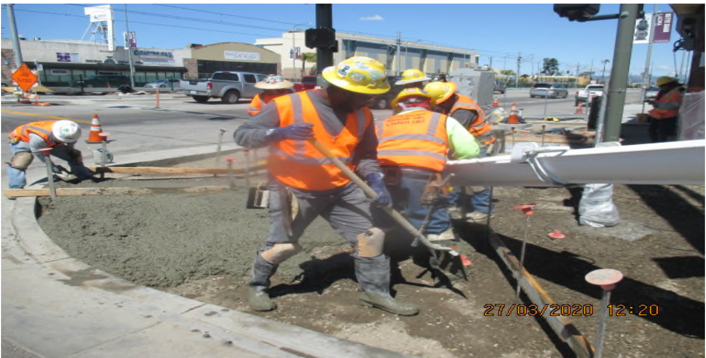
PARK MESA – Placing concrete for new sidewalk and ADA ramp installation on the northeast corner of 54th St and Crenshaw Blvd. 3/27/20
