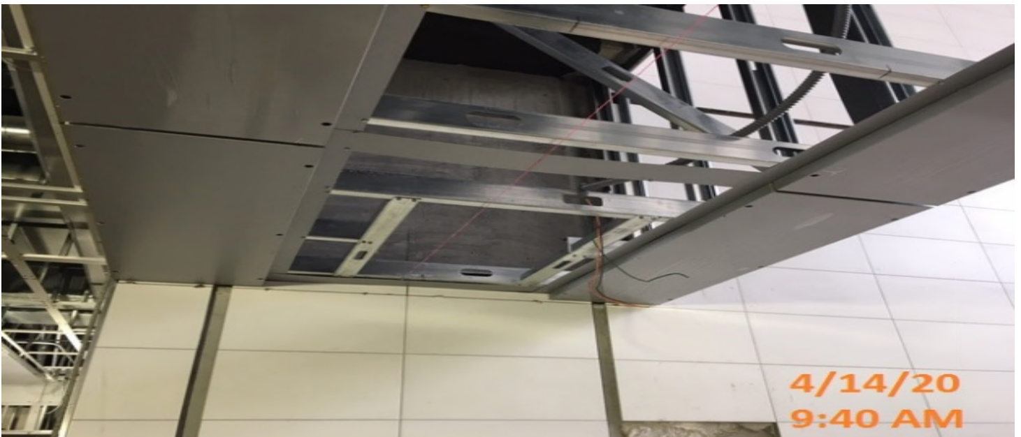
EXPO STATION – Installing light fixtures at the main entrance landing of the concourse level.
