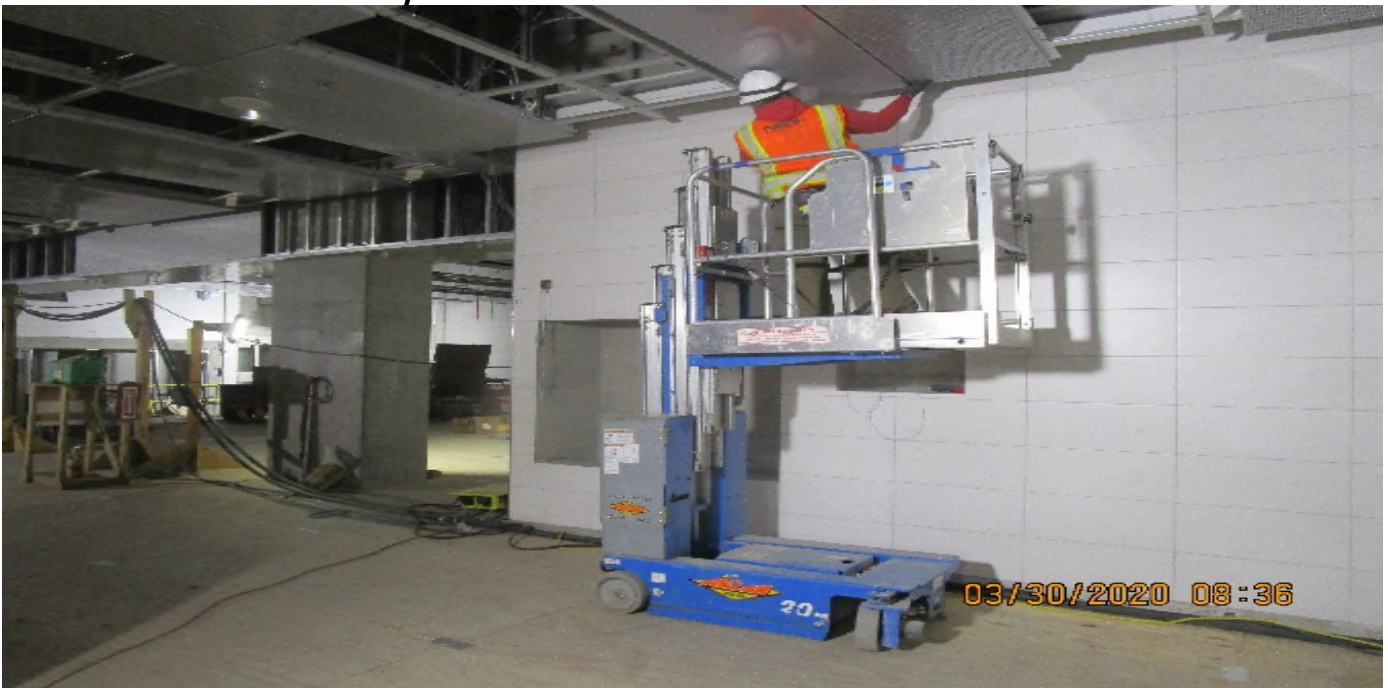
MLK STATION – Continue installing light cove and ceiling panels throughout the Free & Paid Area of the concourse level.
