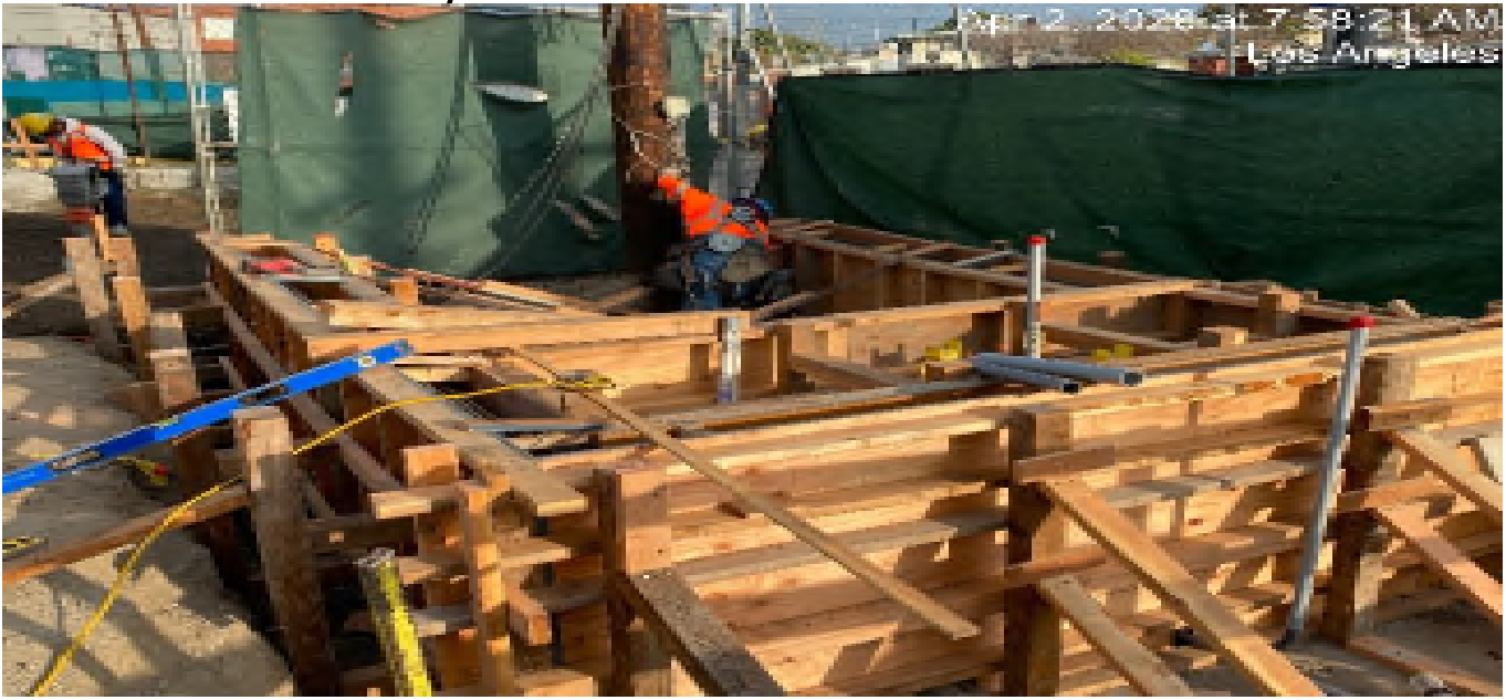
LEIMERT PARK STATION – Continue formwork for the planar wall at the east side of the plaza level.
