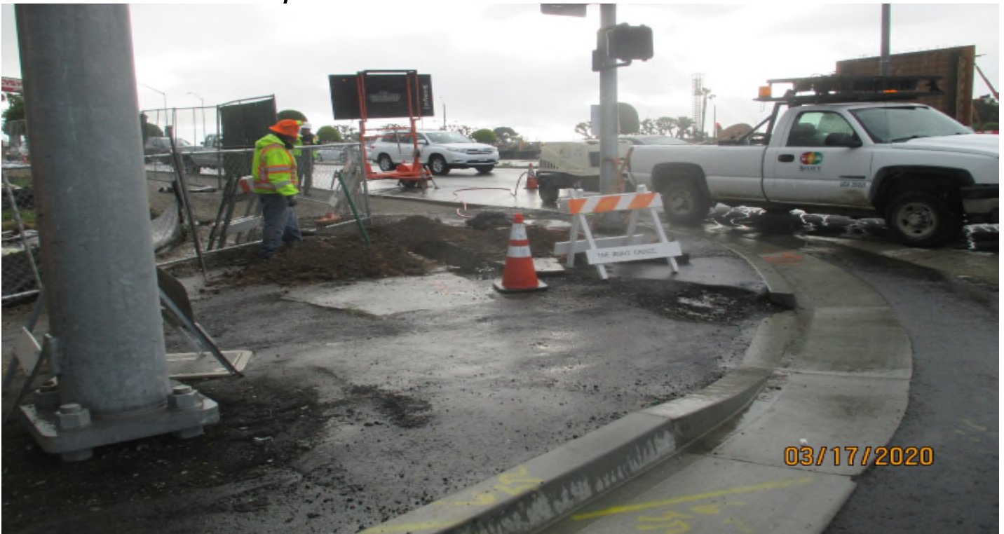
Florence/La Brea – Select Electrical install conduit and a pull box on La Brea. Facing SE.
