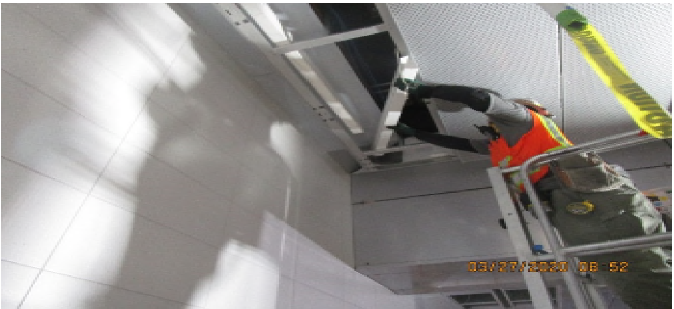
MLK STATION – Continue installing light cove and ceiling panels throughout the Free & Paid Area of the concourse level.
