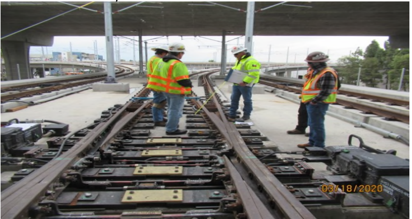
WSSC & Metro WW inspectors at MPF, verifying overall condition of tracks at GL Wye STA 13+90 (looking south)
