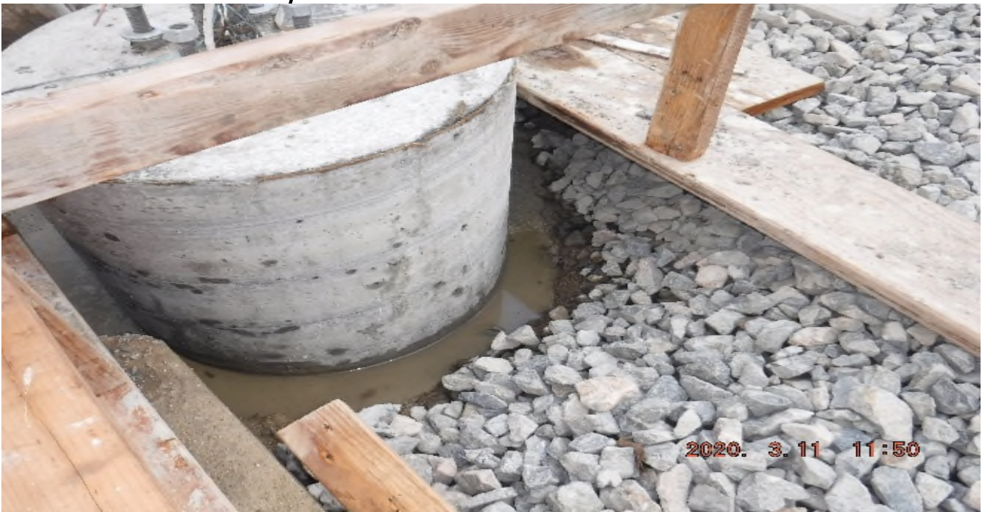
Florence/West – STA 262+80 TK#4. NB looking north – slurry level below finish elevation of sub-grade - water accumulation- PUNCH LIST
