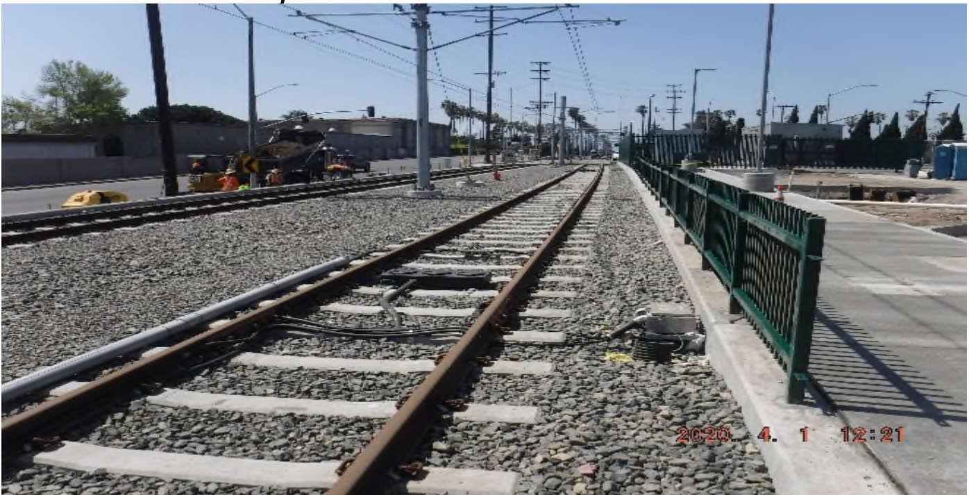
Florence/West – STA 259+00 TK#3-SB looking south – track status; grading work West Station along TK#4 -NBs ballast retainer wall.
