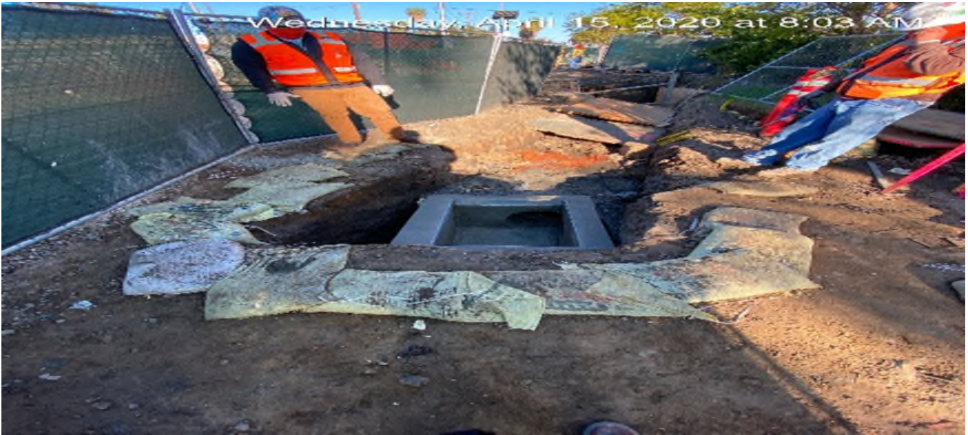
EXPO STATION – Prepping to strip forms for Catch Basin #2 on the northwest section of the plaza.
