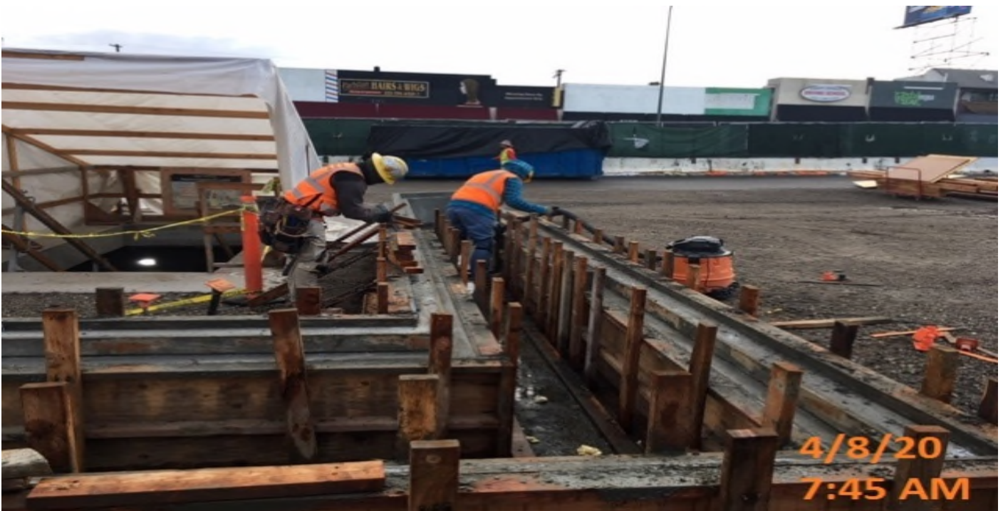
MLK STATION – Stripping forms from the planter wall at the west side of the plaza level.
