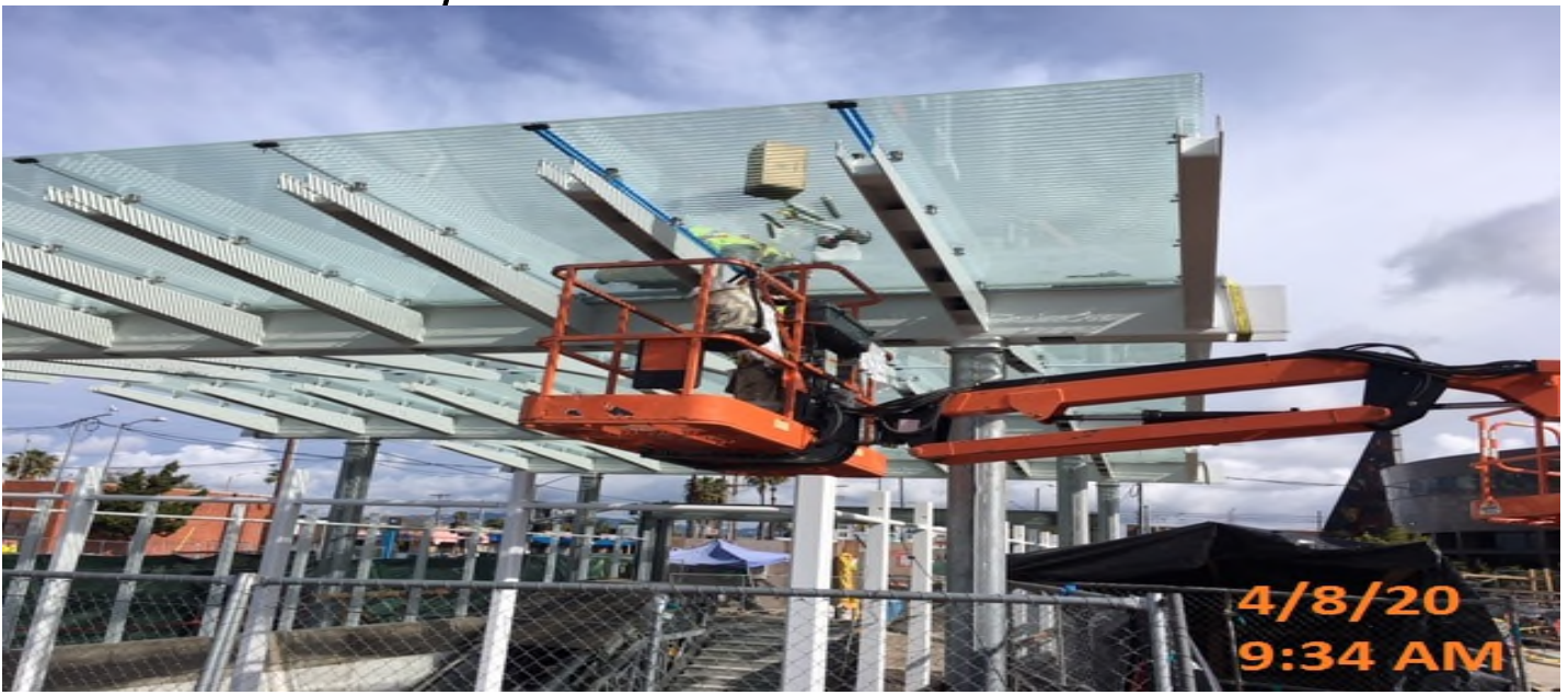
EXPO STATION – Continue caulking glass panel edges with silicone on top of the main entrance canopy at the plaza level.
