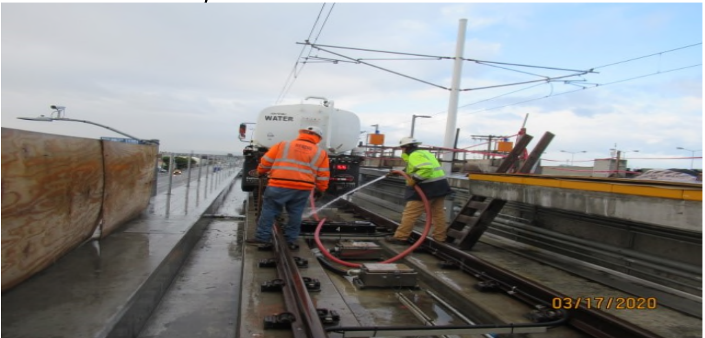
Aviation/Century – HCC on NB #4 track Century. Aviation bridge, using hi-rail water truck to remove excess debris from profile grinder, Work out of Sequence.
