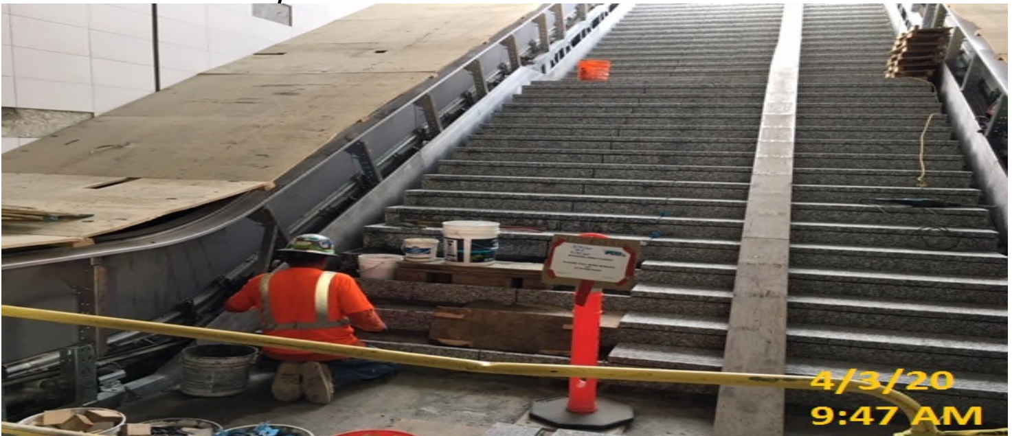
EXPO STATION – Continue installing granite stair treads at the main entrance staircase landing of the plaza level.
