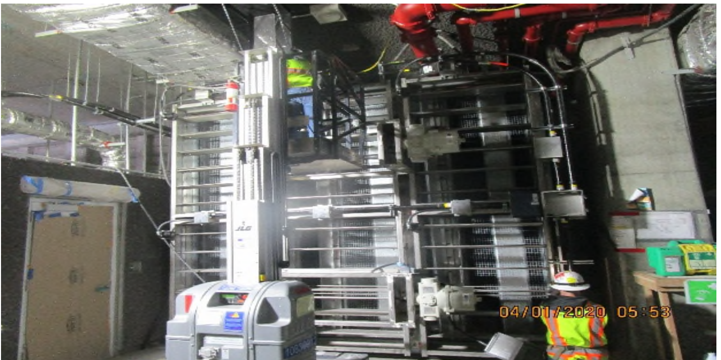
Crenshaw/Vernon - Vernon, Tunnel Vent Plenum (N) #2 C125- TFD-6-352 Continued Nema4X JB`s & 1" FRP to limit switches.
