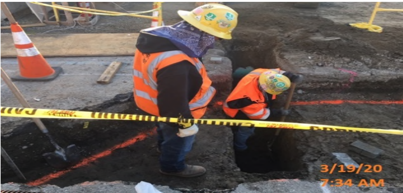
MLK Station - Excavating for 6” pipe for planter wall drainage at the plaza level.
