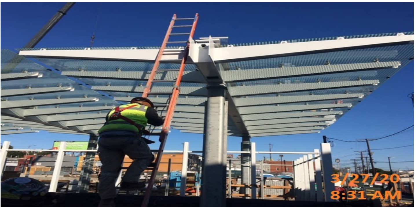
LEIMERT PARK STATION – Finalizing tempered glass installation above the main entrance canopy structure at the plaza level.
