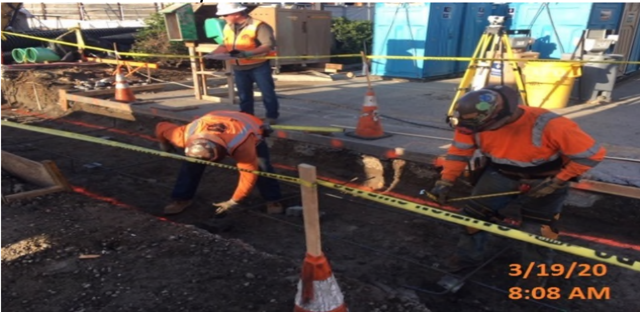
MLK STATION – Began formwork and placing rebar for the planter wall and footings at the west side of the plaza level.
