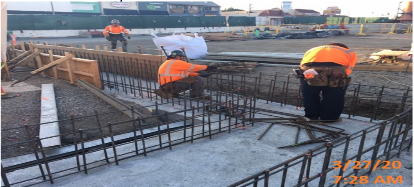
MLK STATION – Continue planter wall and footing installation at the west side of the plaza level.
