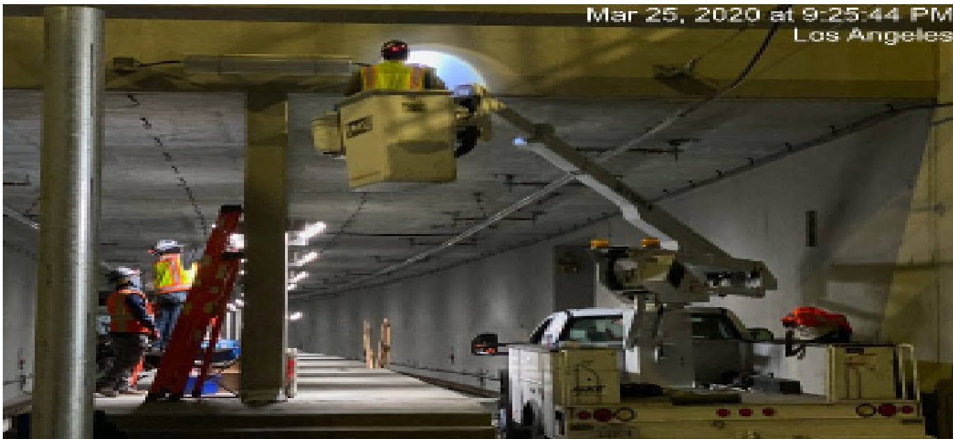
UG-4- Continue pulling wire for the emergency lighting at the south end portal entrance.
