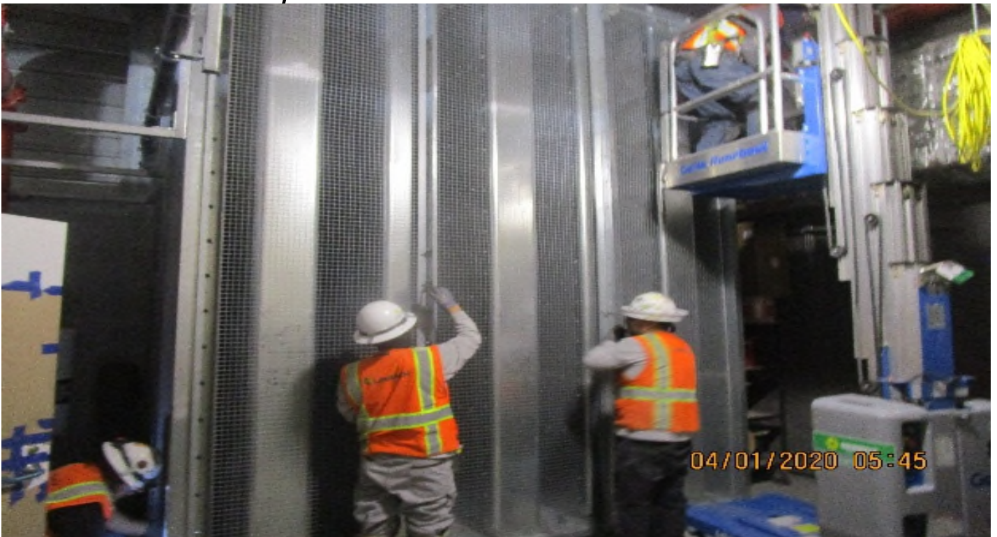
Crenshaw/Vernon - Vernon, Emergency fan room (S) Begin rough in & bolting bird screens prep to install TFD-6-301 per RFI-029.
