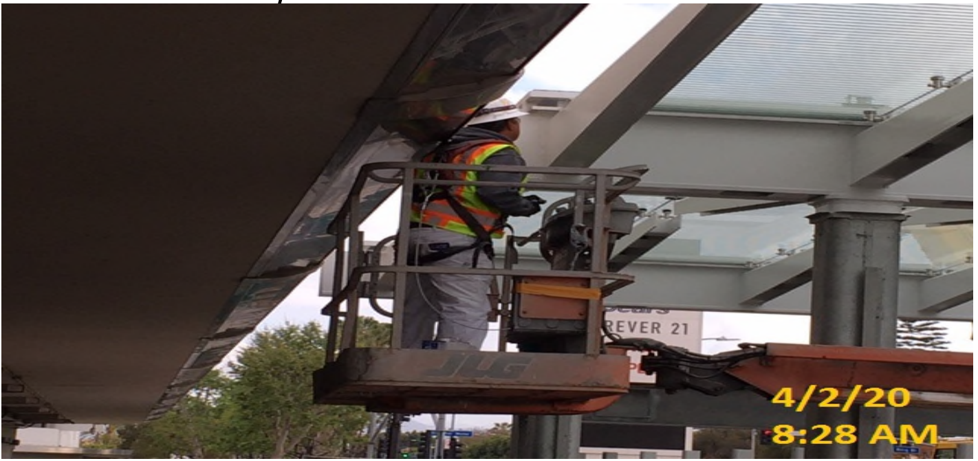
MLK STATION – Continue applying finish coat paint to the main entrance canopy structure at the plaza level.
