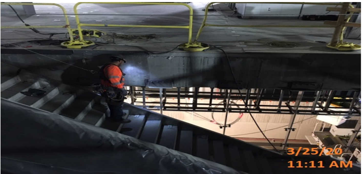
EXPO STATION – Began installing stainless steel cladding panels on the platform ceiling level.
