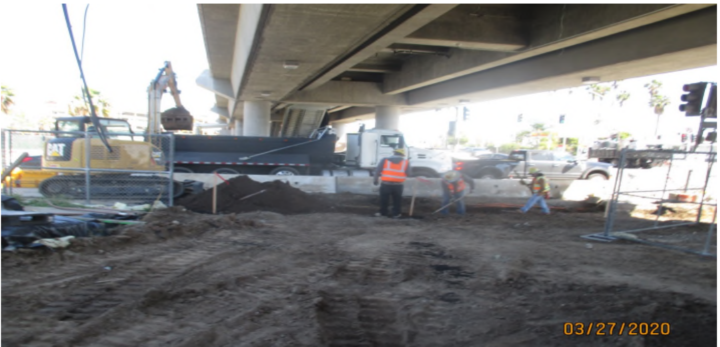
Aviation/Century – Grading for the new curb and gutter on the SW corner of Century and Aviation.
