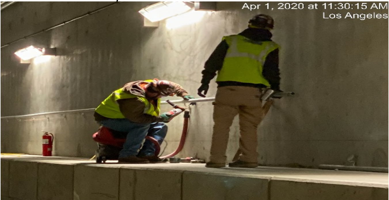
UG3 – Continue installing and welding handrails for the emergency walkway at the northbound tunnel at Sta 300+50.
