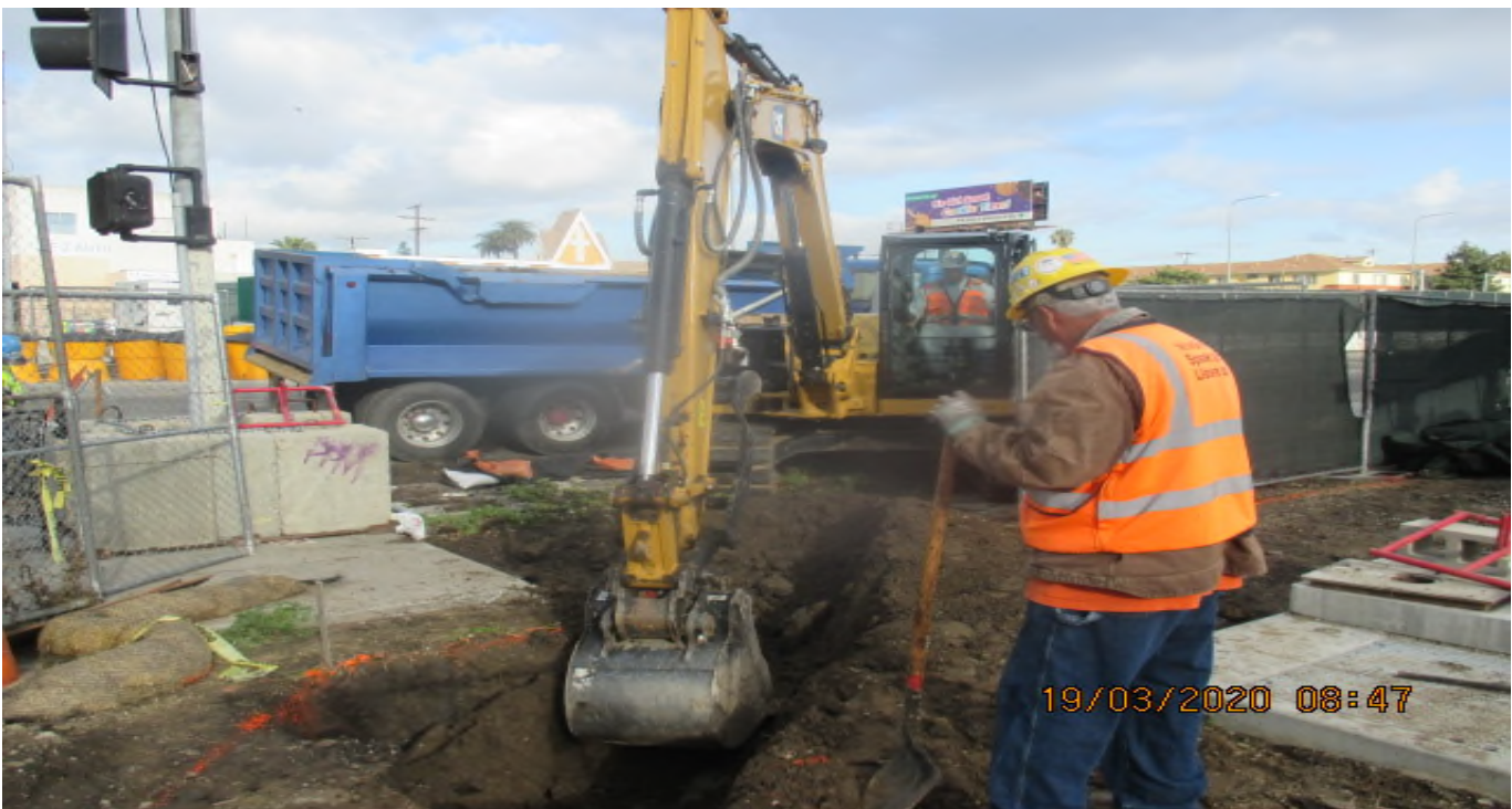
PARK MESA – Excavating for the 12” HDPE storm drain line N-12 at TPSS#7 on 60th St & Crenshaw Blvd. 3/19/20
