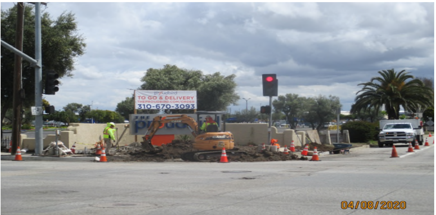
Aviation/Century – Traffic signal and street lighting conduit trenching on 111th and Aviation.
