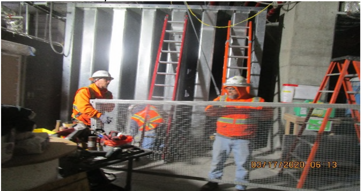
Crenshaw/Vernon - Emergency fan room (N) C142, begin installing bird screens at EVF-6-302 (A)-south attenuator.
