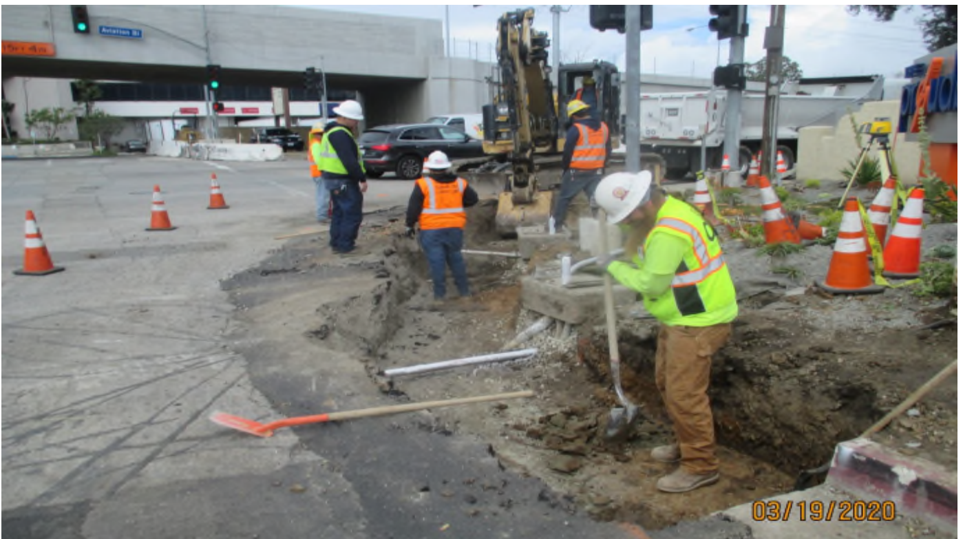
111 th Street – Curb and gutter over excavation on 111th.
