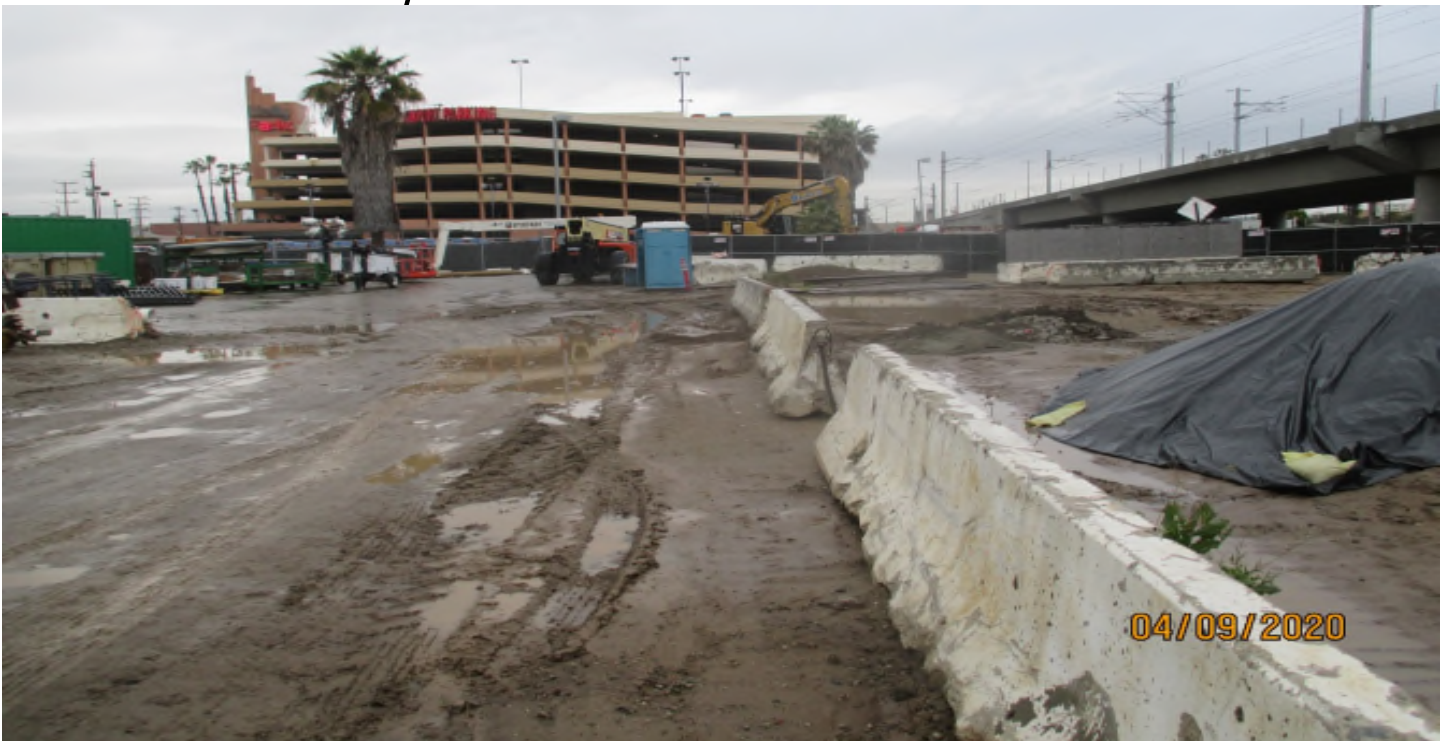
Aviation/Century – Rain damage at Aviation Station.
