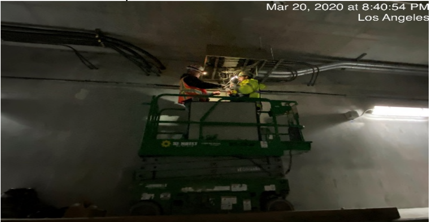
UG-4- Continue splicing wires for the tunnel booster junction boxes at the southbound tunnel at Sta 374+00.
