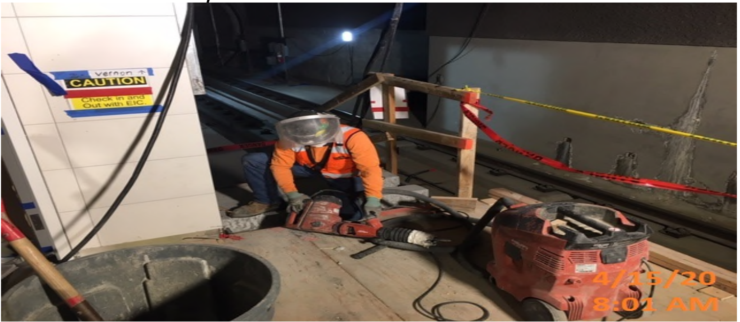
MLK STATION – Preparing for end gate installation at the northbound stair landings of the north end of the platform level.
