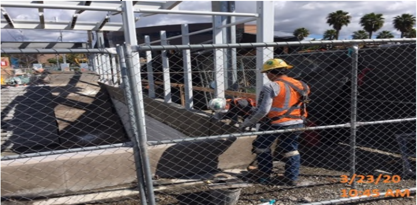
EXPO STATION – Continue surface finishing the wind screen curbs around the main entrance of the plaza level.
