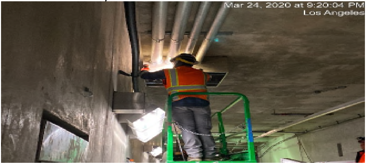
UG-4- Continue splicing and grounding wires for the tunnel booster junction boxes at the southbound tunnel at Sta 374+00.
