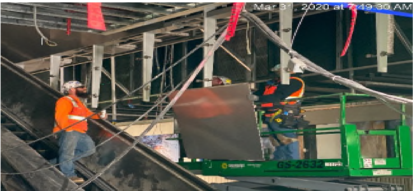
LEIMERT PARK STATION – Continue installing stainless steel cladding panels on the platform ceiling level.
