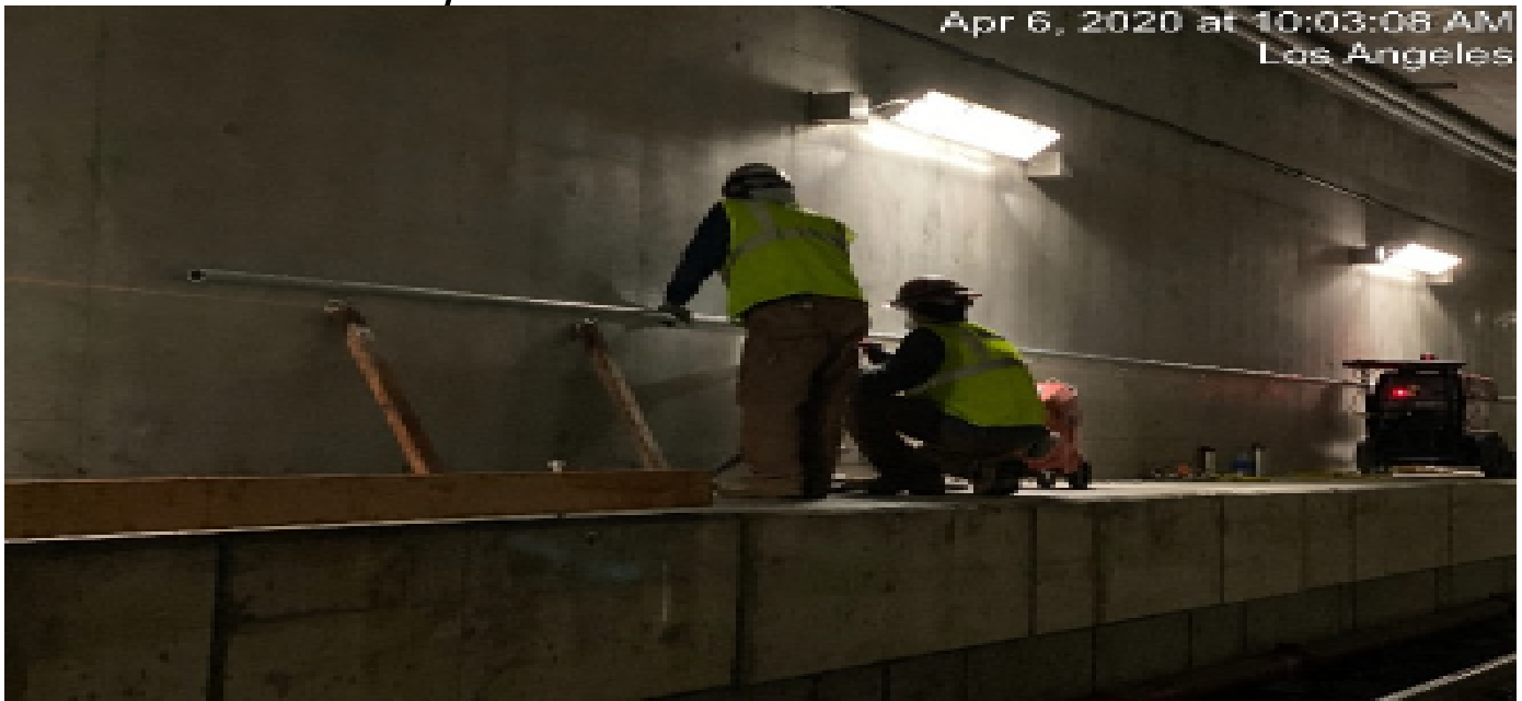
UG3 – Continue installing handrails for the emergency walkways on both the north and southbound tunnels.
