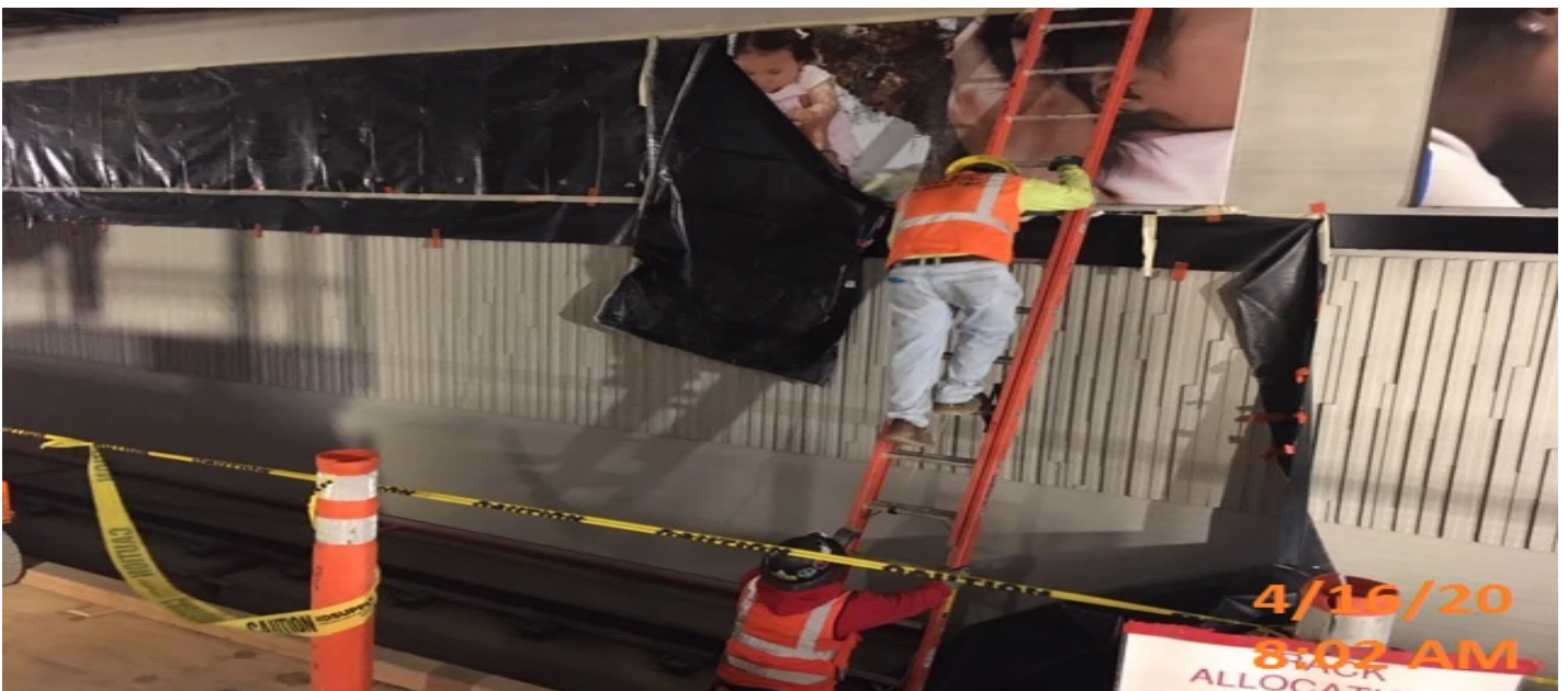
MLK STATION – Removing protective wrap for artwork inspection at the platform level.
