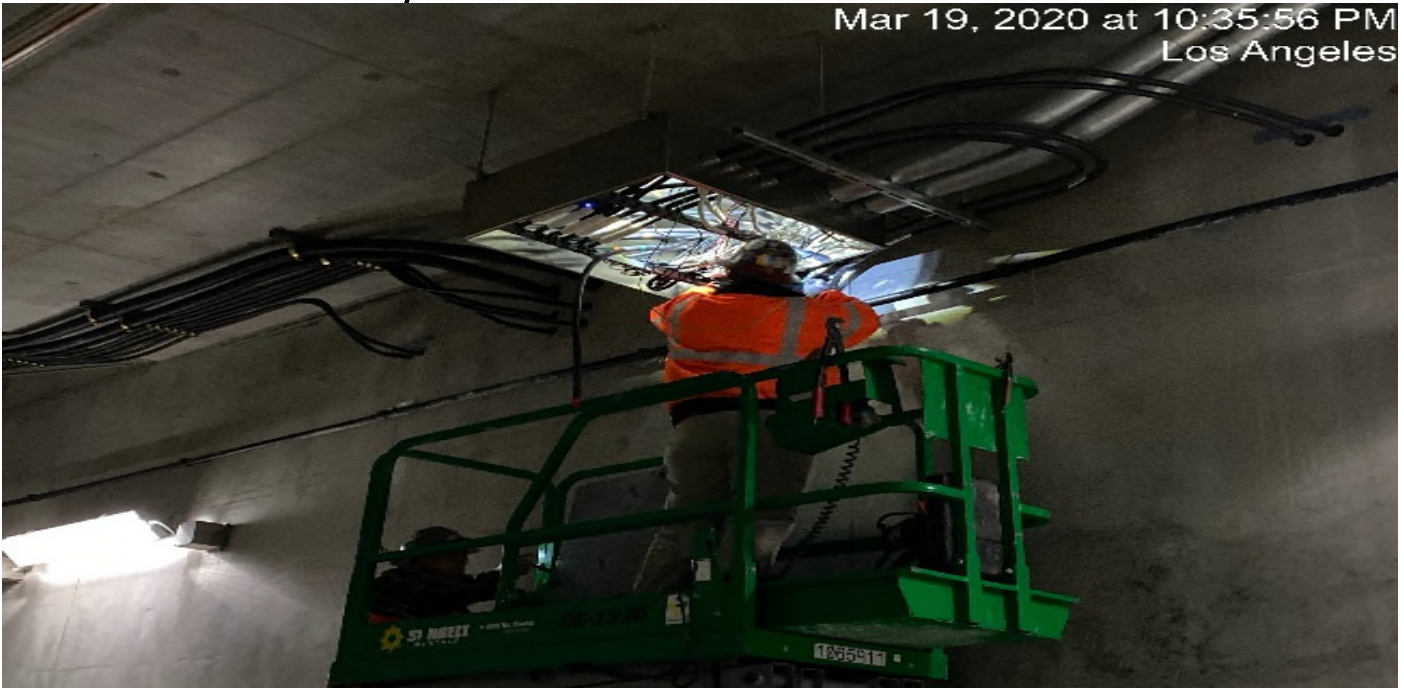
UG3 – Continue splicing wires for the tunnel booster junction boxes at the southbound tunnel at Sta 291+50.
