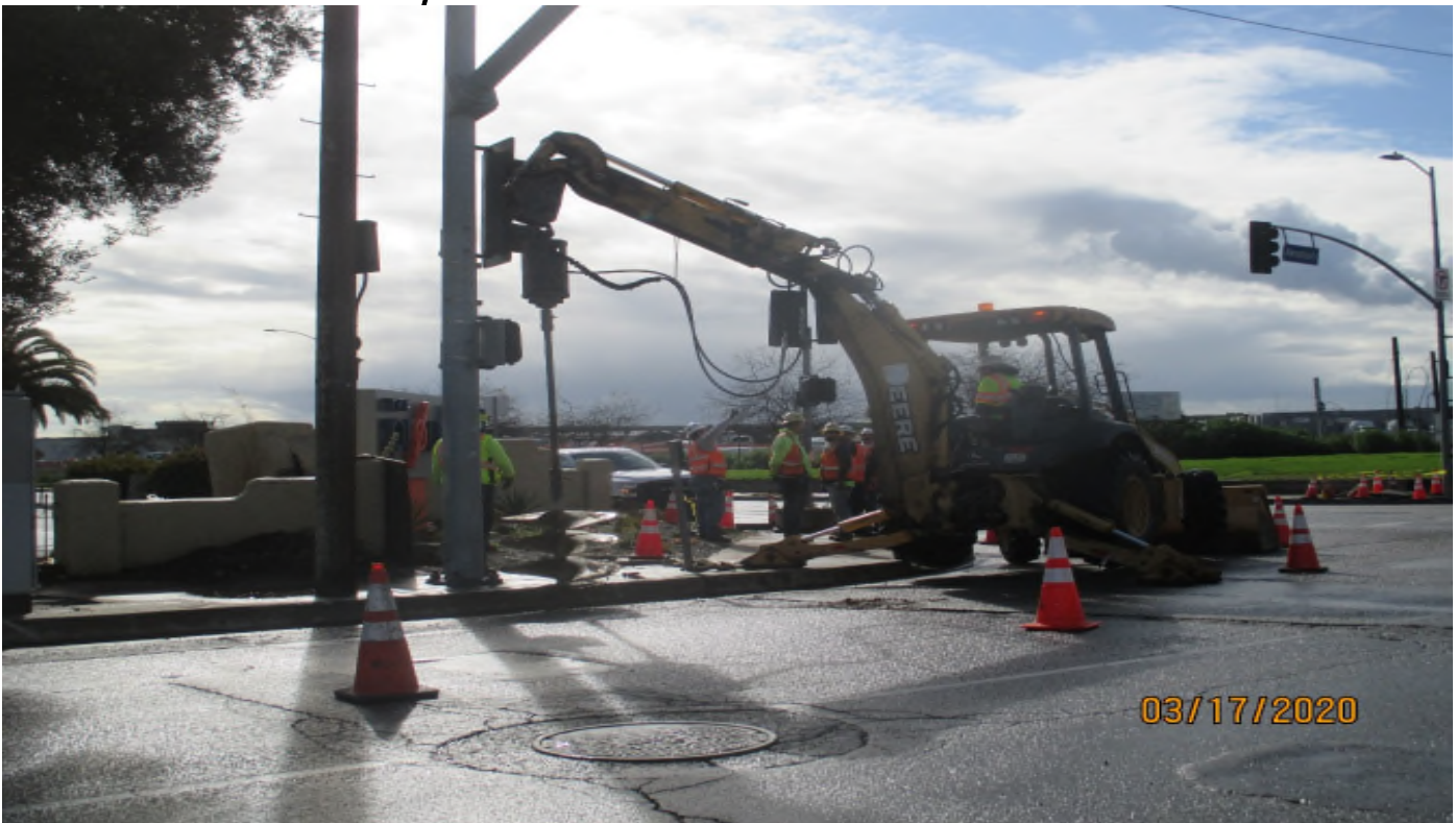
Aviation/Century – Auguring for a traffic signal foundation on the NE corner of 111th & Aviation. Facing SE.
