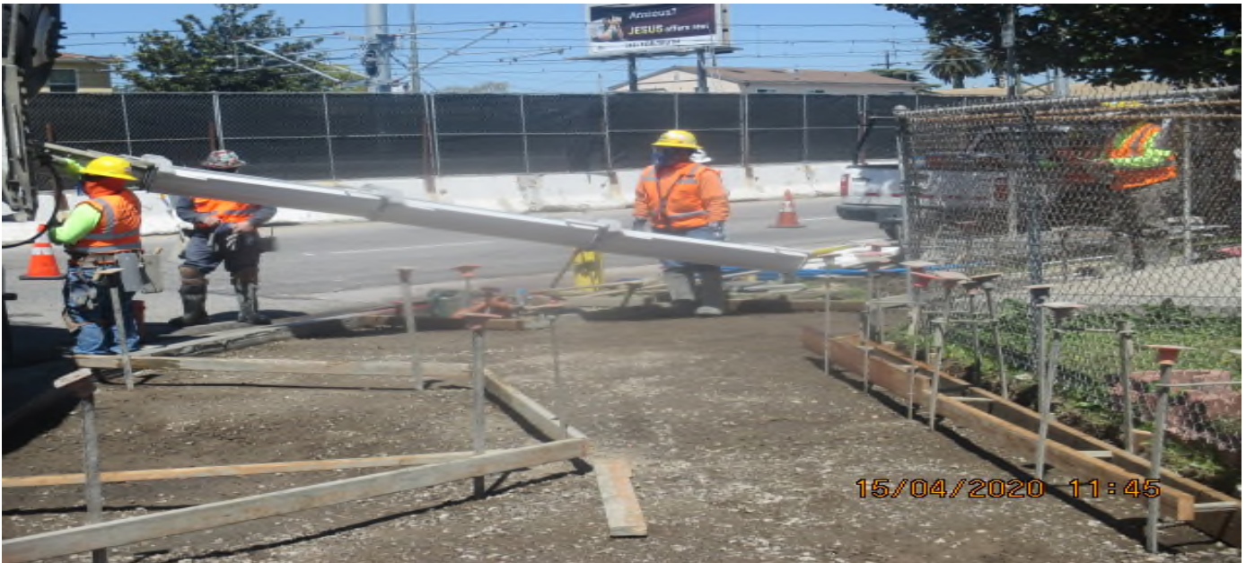
PARK MESA – Placing concrete for the new sidewalk and ADA ramp installation on the northeast corner of 59th Pl & Crenshaw Blvd. 4/15/20
