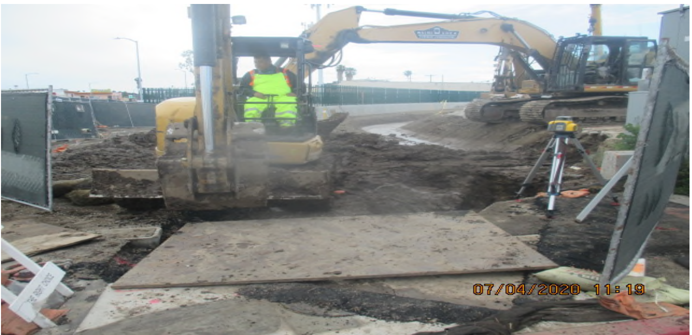
UG3 – Continue excavating for 18” HDPE drain line connection to Catch Basin #1 on the southwest corner of 67th St and Crenshaw Blvd. 4/7/20
