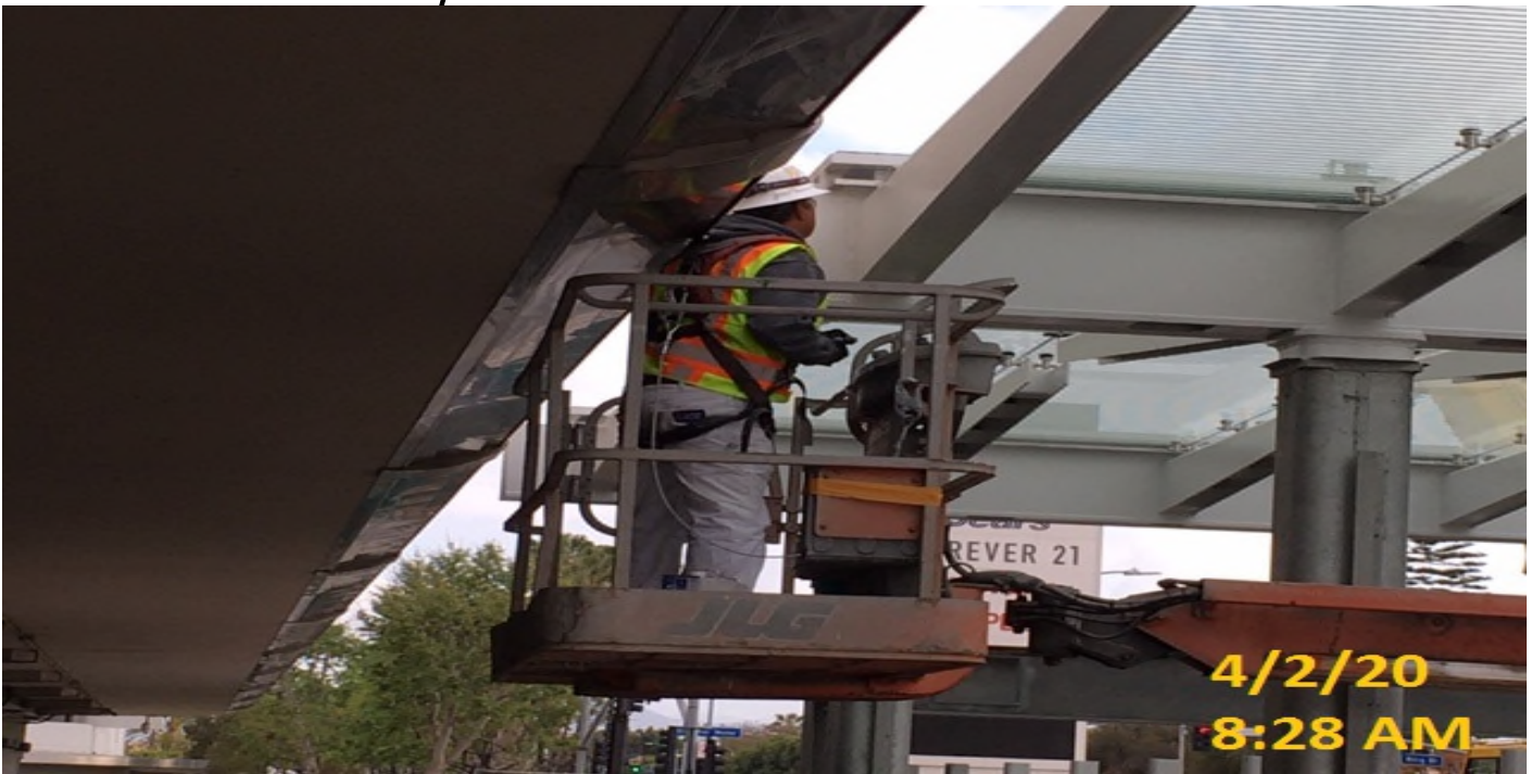
Crenshaw/MLK - MLK – Mariscal Painting applying 1st coat of finish touch up to main entrance canopy.
