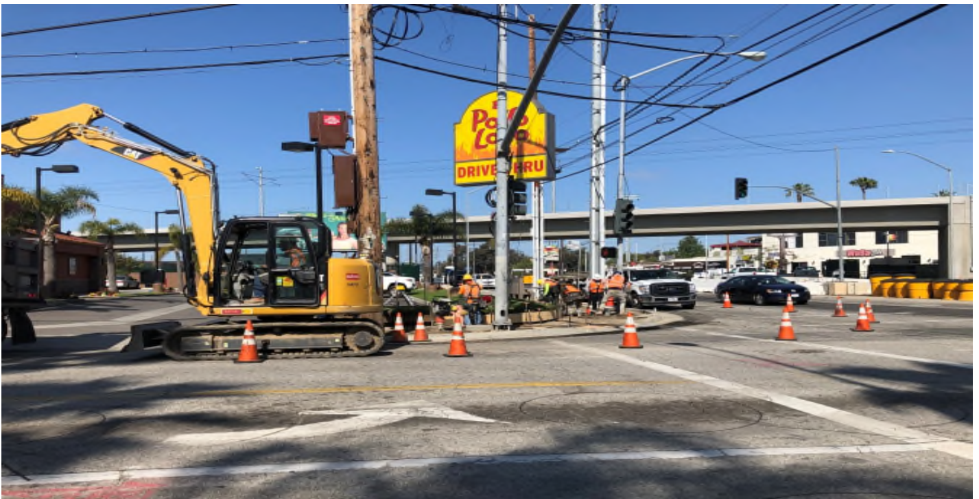
Manchester Bridge – Setting forms for the ADA ramp at Aviation and Manchester.
