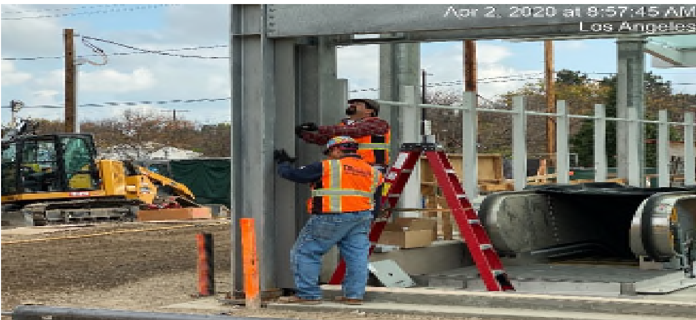
LEIMERT PARK STATION – Began installing overhead coiling grille components to the main entrance canopy at the plaza level.
