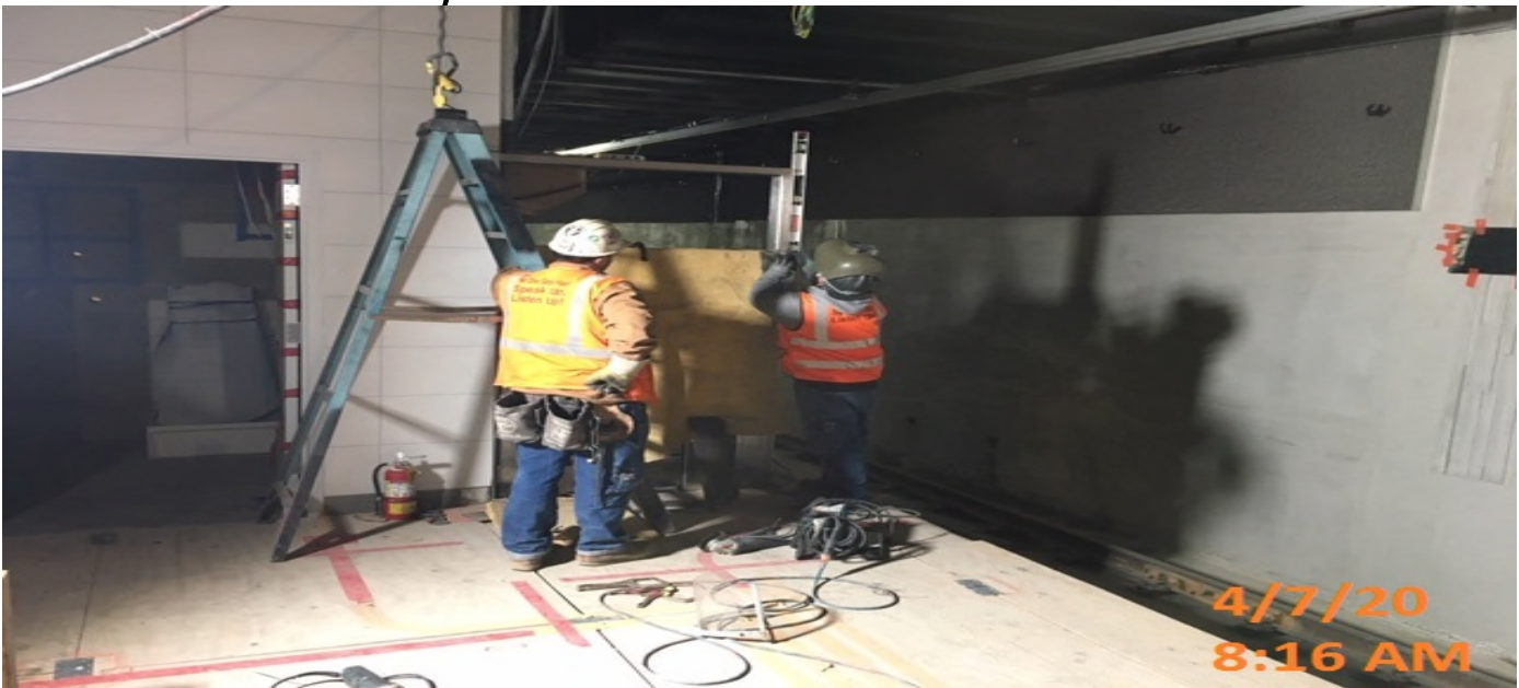
EXPO STATION – Continue end gate installation for both the north and southbound stair landings on the south end of the platform level.
