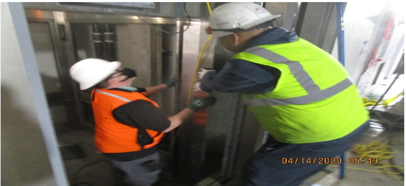
MLK STATION – Began cab door stop installation for all the Elevators at the concourse level.
