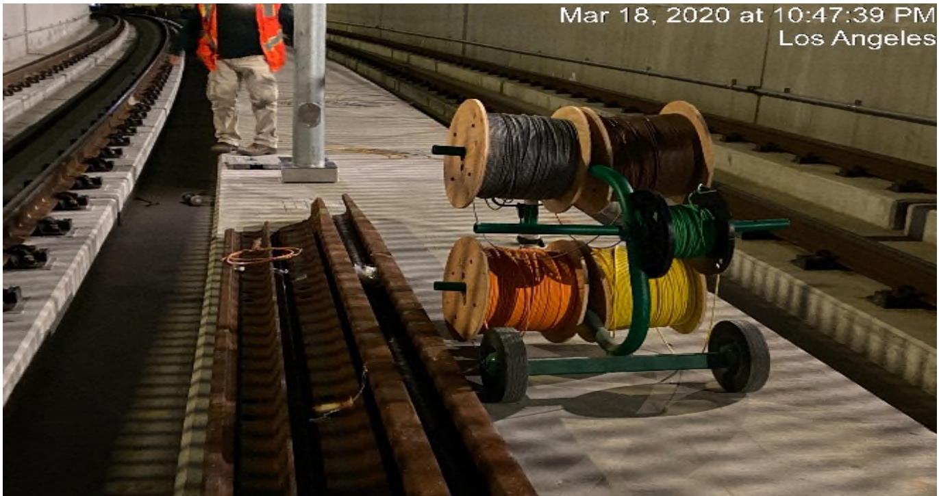
UG-4- Continue pulling wire for the pole lighting at the south end portal entrance.
