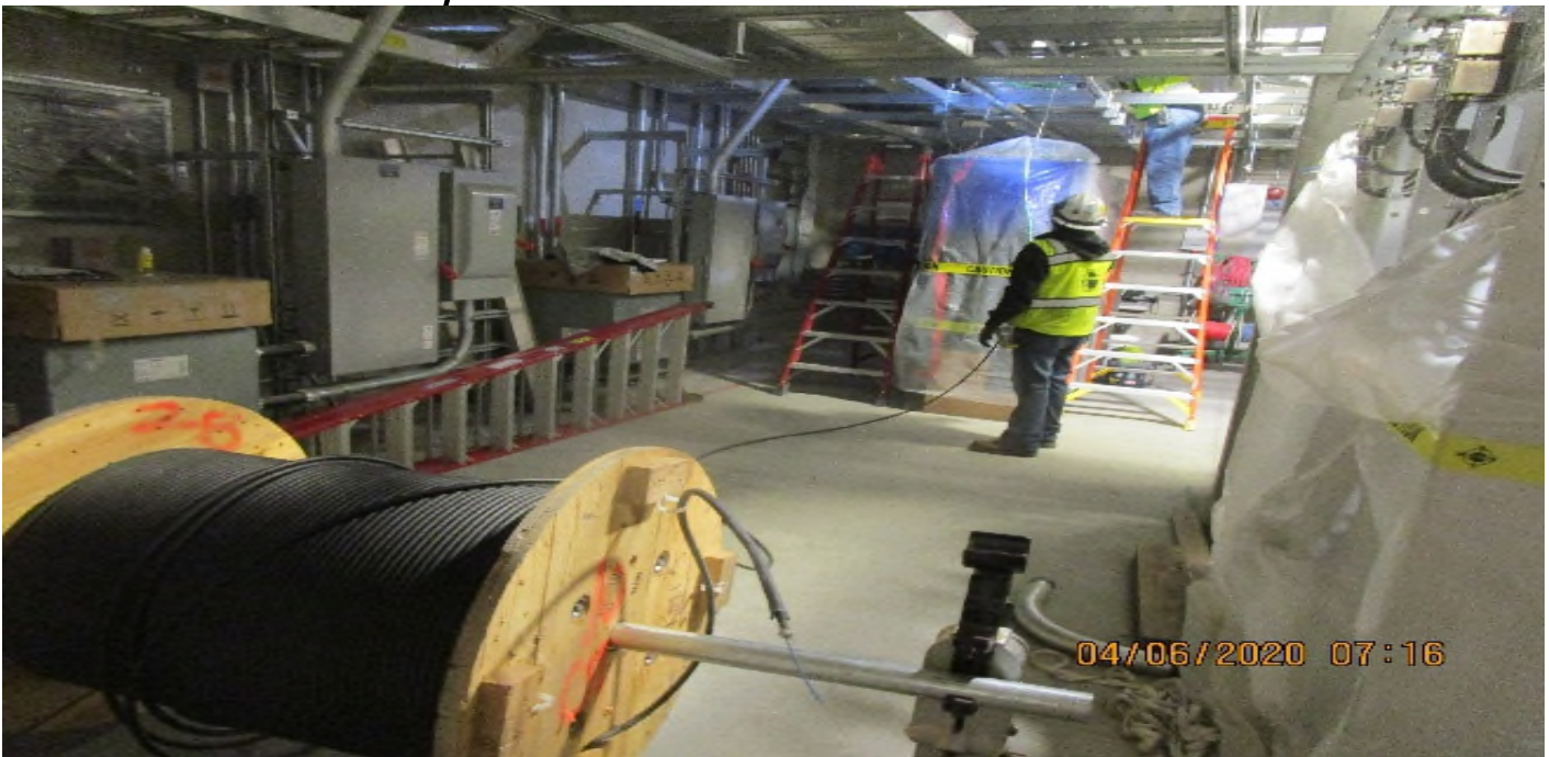
Crenshaw/MLK - MLK, TC&C Room C113, begin pulling 12-SM fiber optic cable from MDF-3 to RIO-03 in Aux power room (S) C109.
