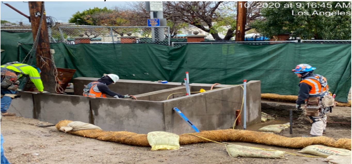
LEIMERT PARK STATION – Setting string lines in preparation for formwork for the planter section stair risers at the plaza level.
