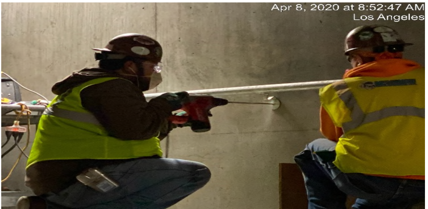
UG3 – Continue installing handrails for the emergency walkways on both the north and southbound tunnels.
