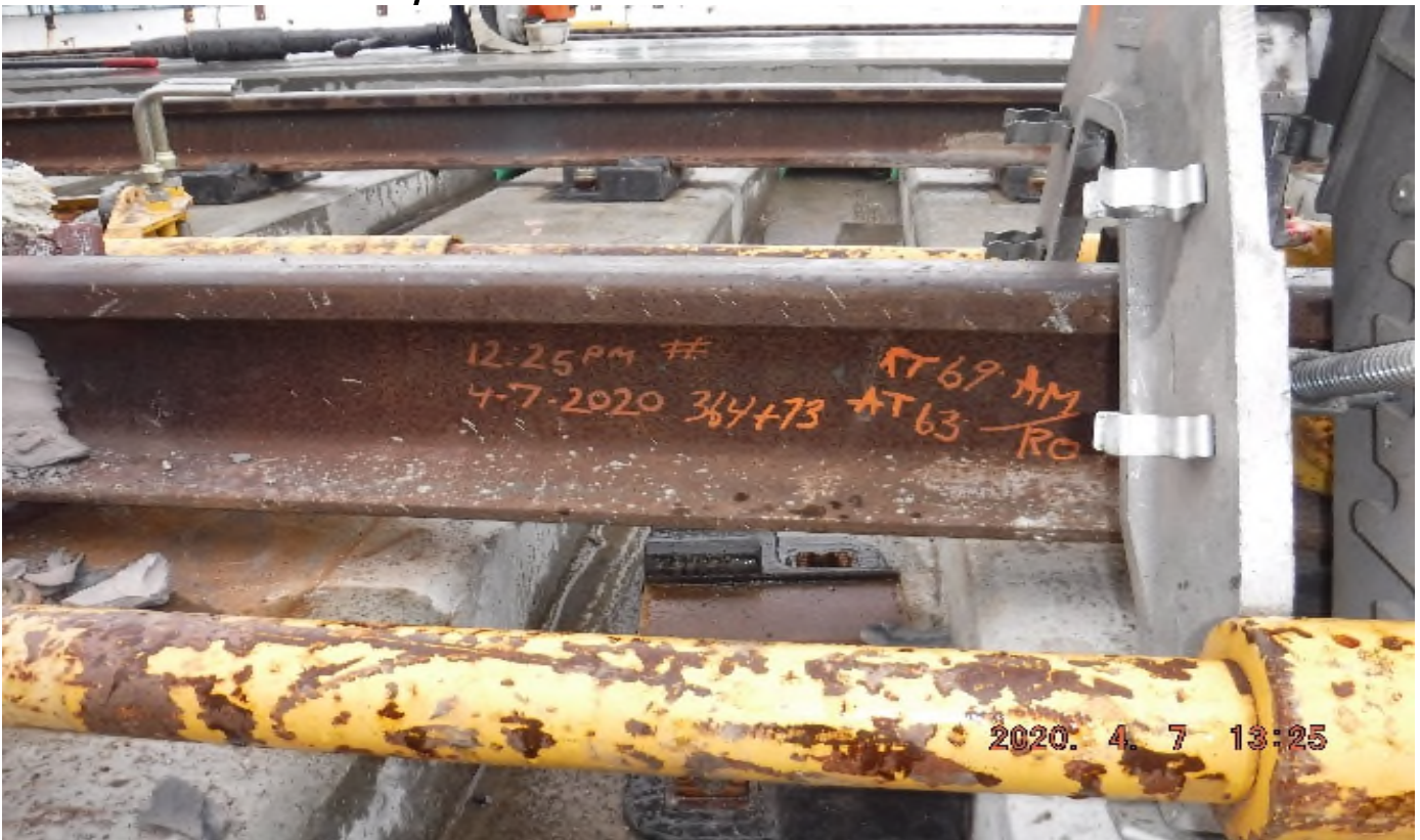
48 th Street - STA 364+73 TK#3-SB looking east – left rail de-stress weld (48th St)
