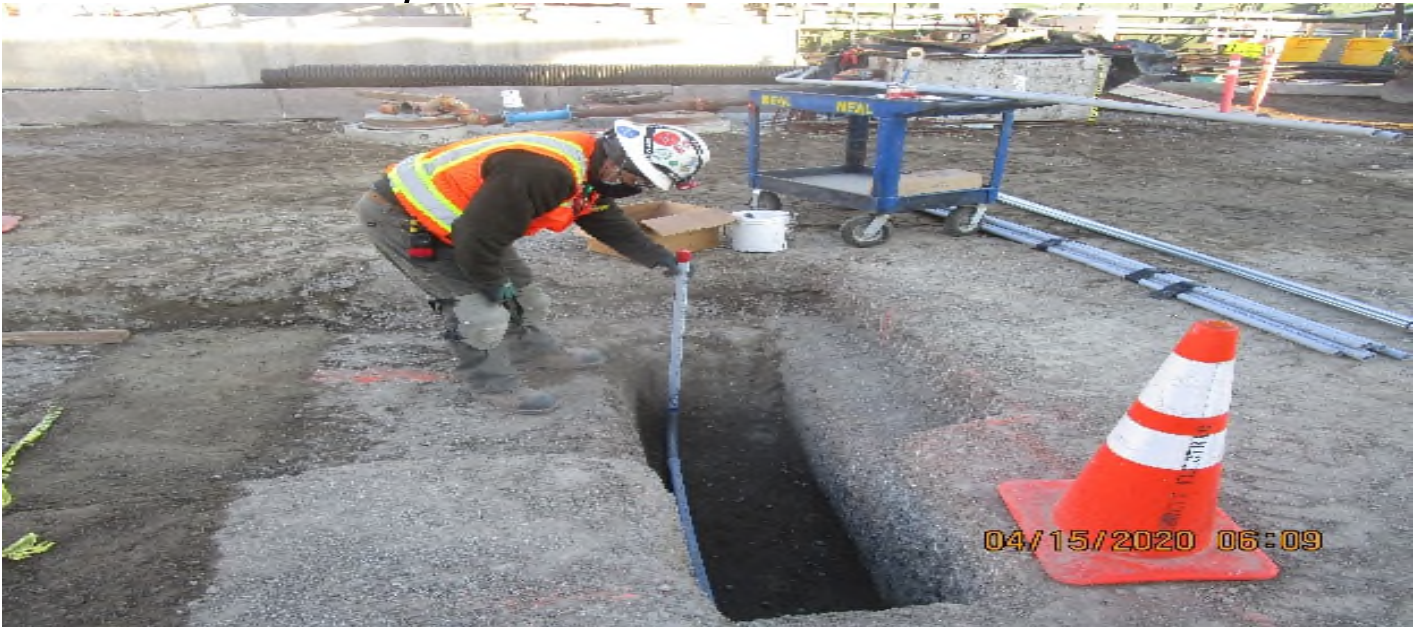
LEIMERT PARK STATION – Begin rough-in of PVC pipe for the free standing map case installation at the plaza level.
