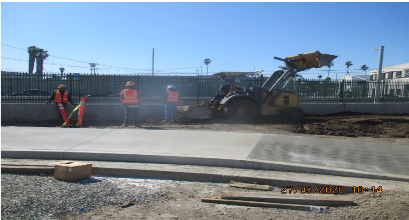
UG3 – Continue grading and excavating for the culvert drainage along the southbound barrier wall in preparation for concrete placement. 3/27/20
