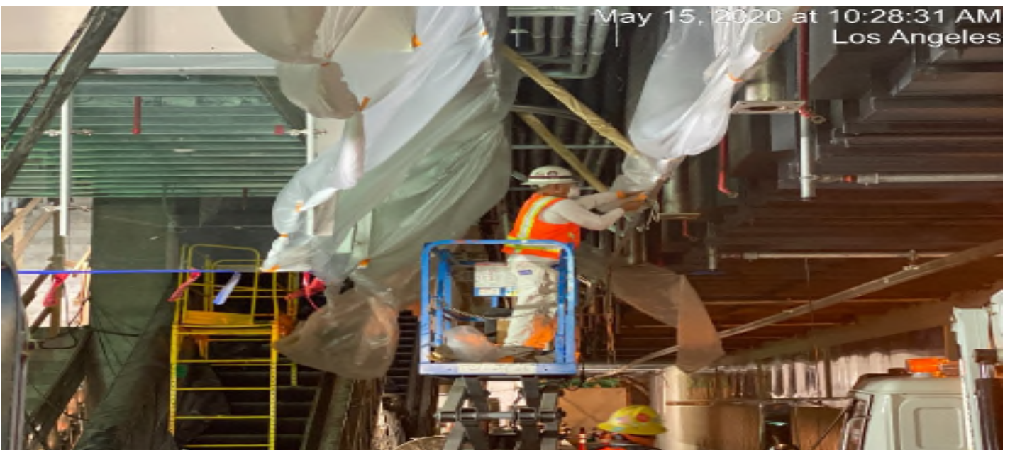
LEIMERT PARK STATION – Preparing for primer application to the ceiling conduits at the platform level.
