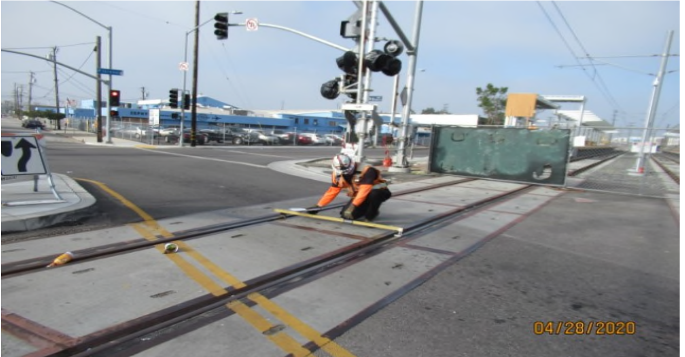
Florence/Hindry – WSCC QC track inspector verifying cross level on #4 NB track at Hindry grade crossing for BIM360 inturnal punch list updates (looking southeast)
