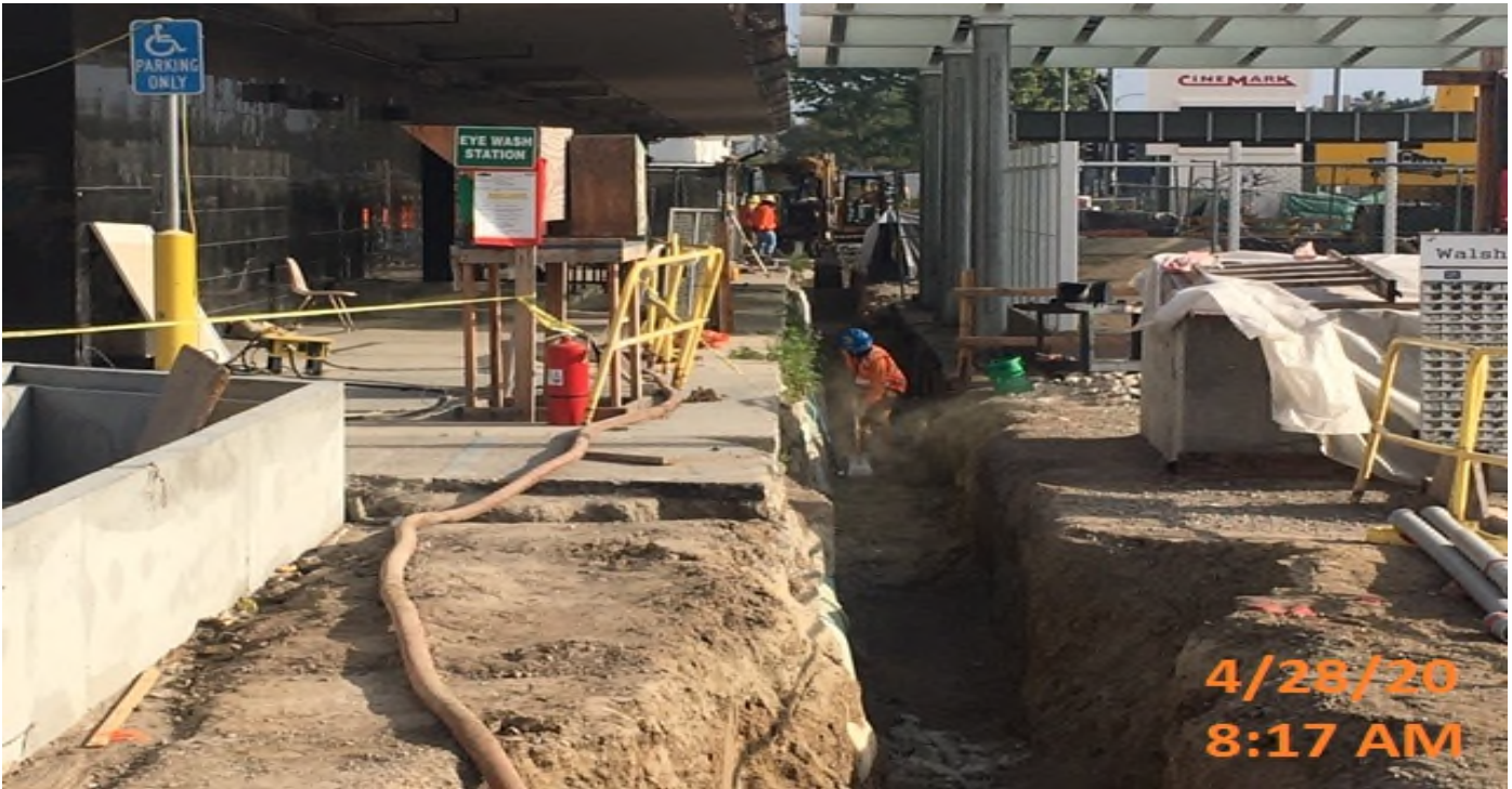
MLK STATION – Continue excavating for new 12” HDPE drainage pipe adjacent to the main entrance canopy structure at the plaza level.
