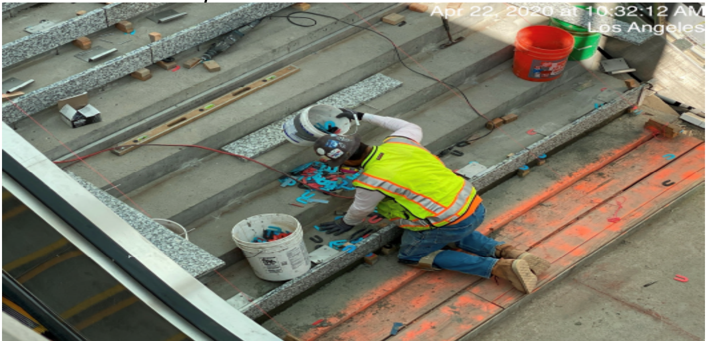
LEIMERT PARK STATION – Continue granite thread and riser installation at the main stair case landing of the plaza level.
