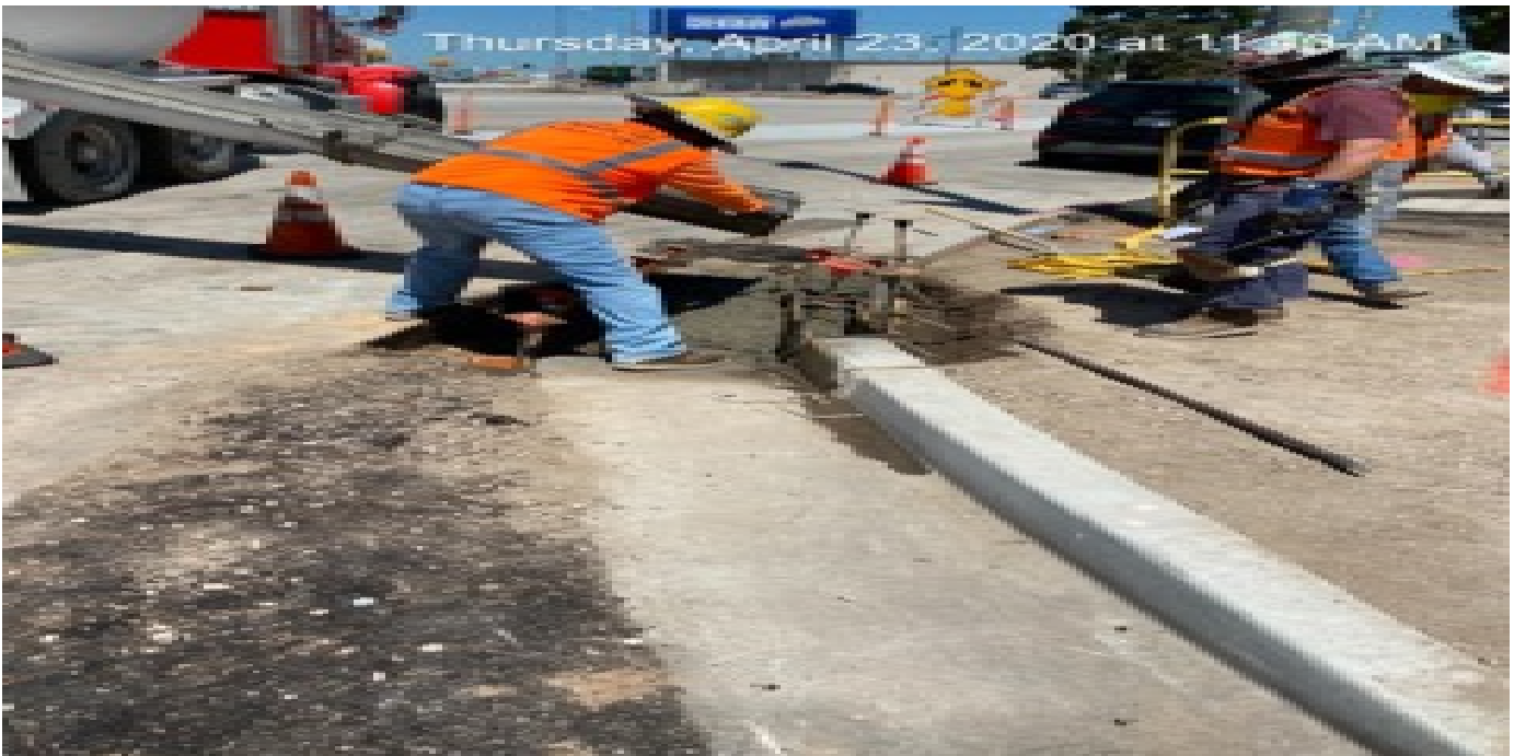
LEIMERT PARK STATION – Placing concrete for new curb/gutter on the south and northeast corners of 46th St and Crenshaw Blvd.
