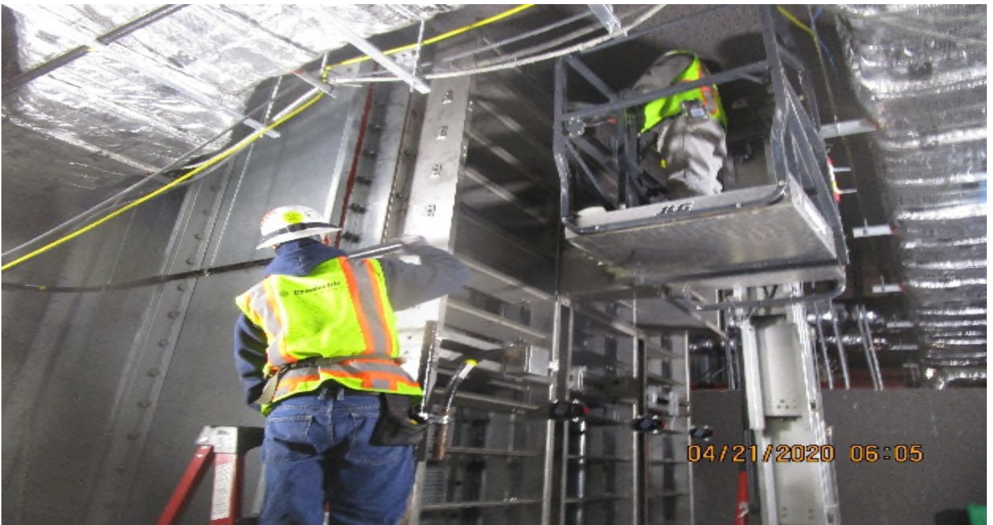
Crenshaw/Vernon - Vernon Concourse, Tunnel vent plenum (S) C106, TFD-6-101 continued rough 1" FRP at actuators & limit switches.
