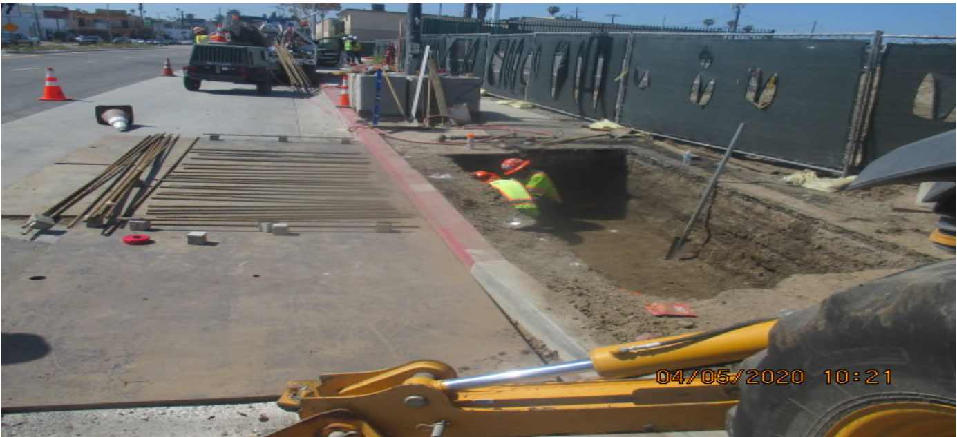
UG3 – Installing rebar mat for the street light foundation on the southwest corner of 67th St and Crenshaw Blvd. 5/4/20
