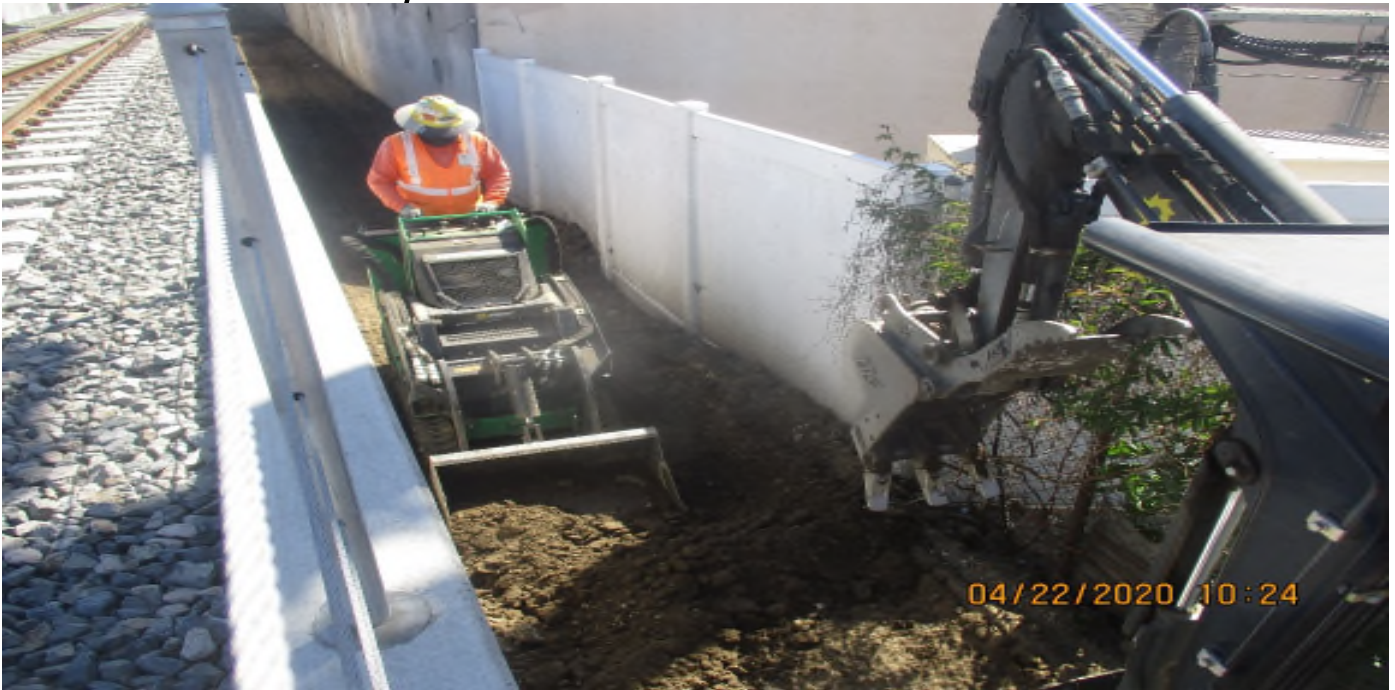
Florence/West – WSCC Continue grading for swale area at West Station ballast wall.
