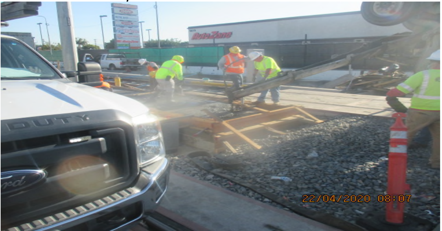
Hyde Park Station – Placing concrete for the south end entrance ramp at the platform. 4/22/20
