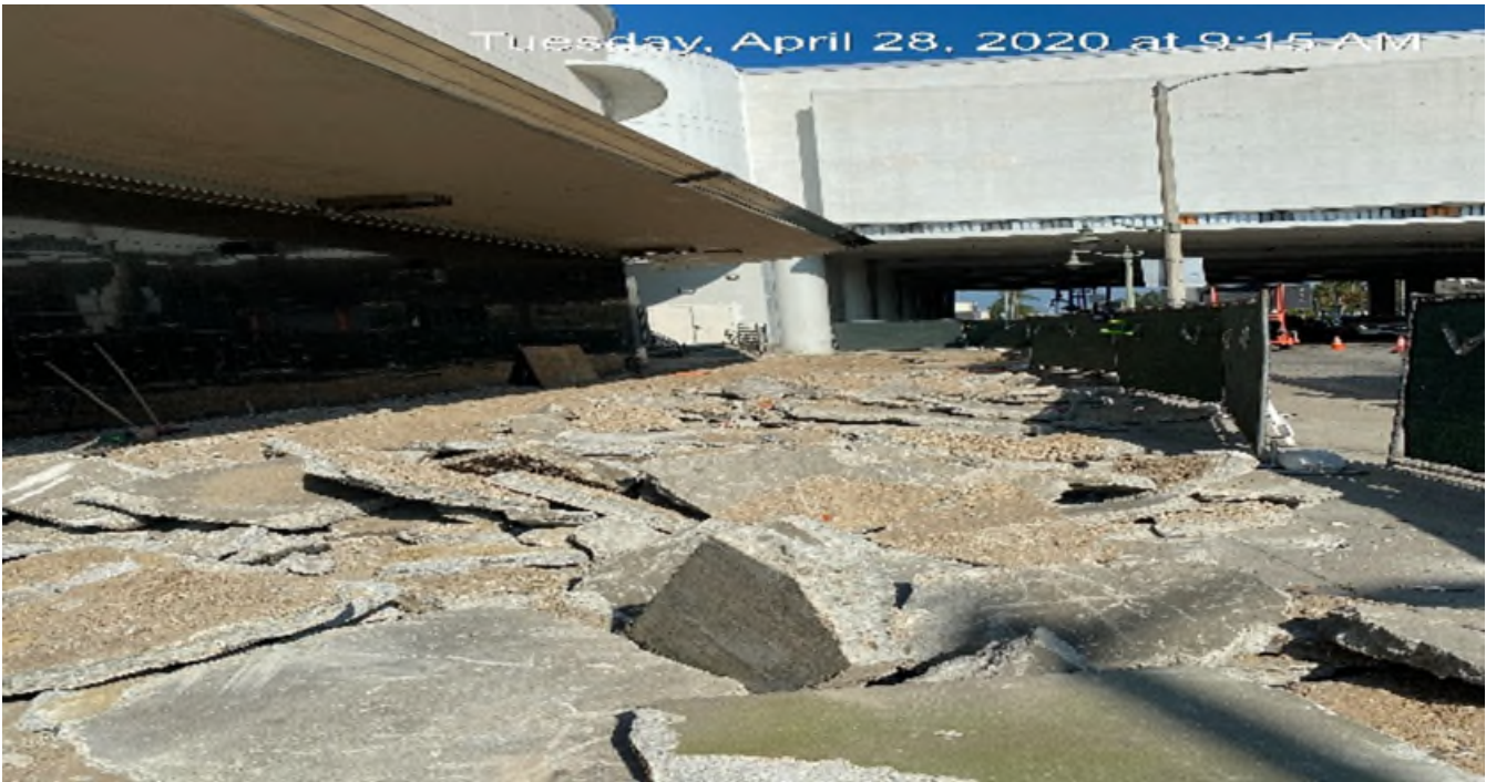
MLK STATION – Continue excavation/demolishing of the eastbound sidewalk on the northwest corner of the plaza.
