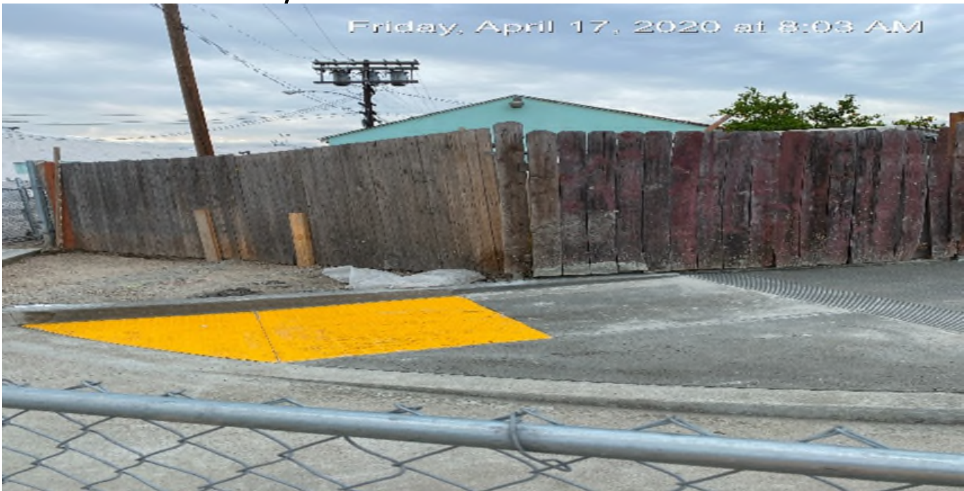
EXPO STATION – Finalized the new ADA ramp installation on Bronson Ave east of the plaza.
