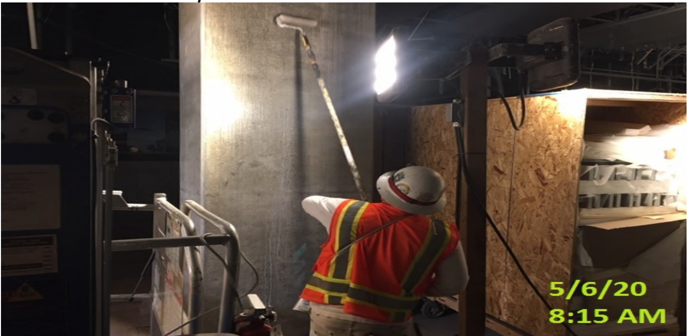
MLK STATION – Applying sealer prior to anti-graffiti finish coat to all the columns at the platform level.
