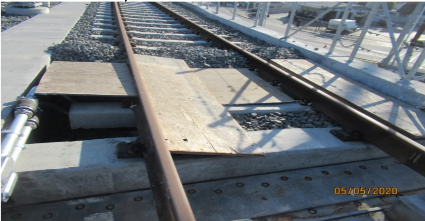
Manchester Bridge - Manchester Bridge NB #4 track STA 121+45 no condition changes for disturbed ballast on Metro's Punch list, item #250 in Segment A
