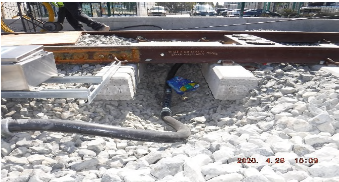
57th STREET- STA 329+75 TK#4 , NB looking east – checking depth of system conduit imbedded in track structure south of 57th St – PUNCH LIST
