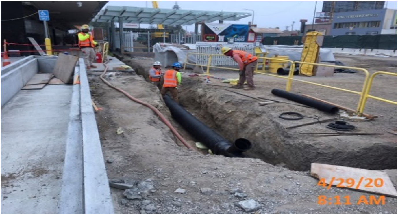
MLK STATION – Installing 12” HDPE drainage pipe on the west side of the plaza level.
