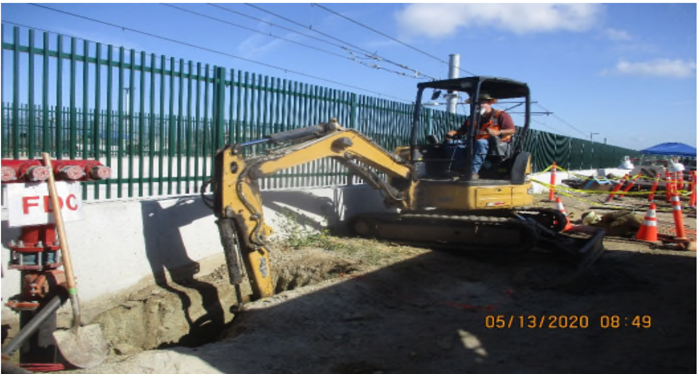
AVIATION/CENTURY - WSCC Excavation for Fire line at SB Aviation at end of UG-1
