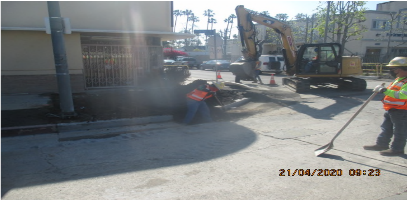
LEIMERT PARK STATION – Excavating for new sidewalk and ADA ramp installation on the northeast corner of 46th St and Leimert Blvd. 4/21/20
