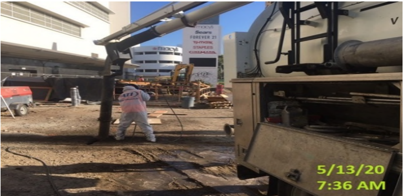
MLK STATION – Continue potholing for upcoming tree well installation throughout the plaza level.
