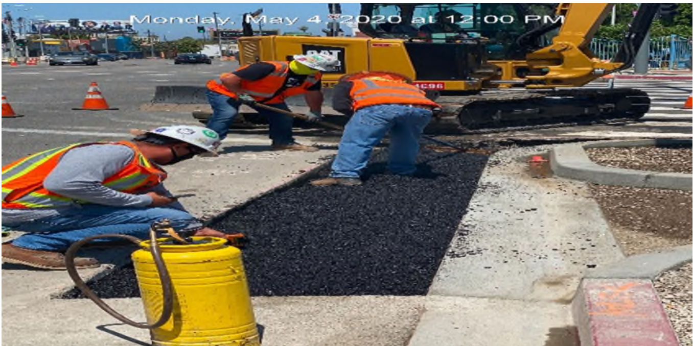
LEIMERT PARK STATION – Placing asphalt concrete around the curb/gutter on the southeast corner island of Vernon Ave and Crenshaw Blvd.
