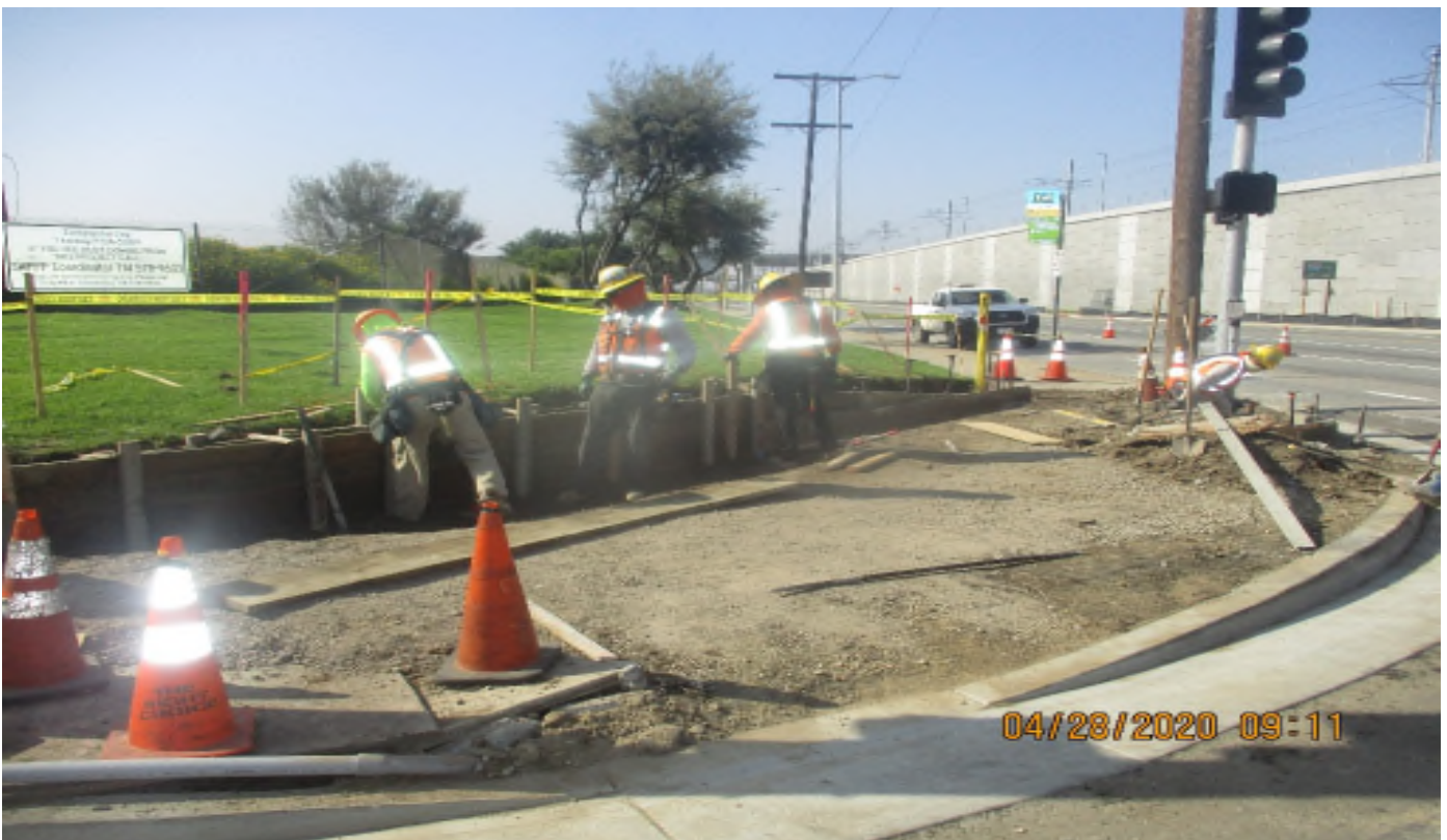
Aviation/Century – WSCC Form and place concrete for small retaining wall at S/WCOR of 111Th and Aviation.
