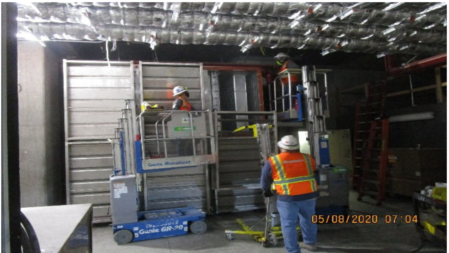
MLK STATION – Installing damper sections and began actuator layout for TFD-7-122 in the North Emergency Fan Room C – 142 of the concourse level.
