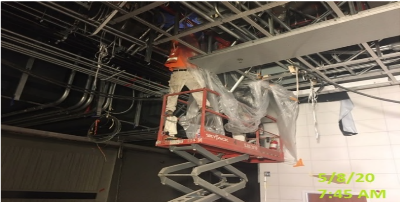
MLK STATION – Preparing for primer application to the ceiling conduits at the platform level.
