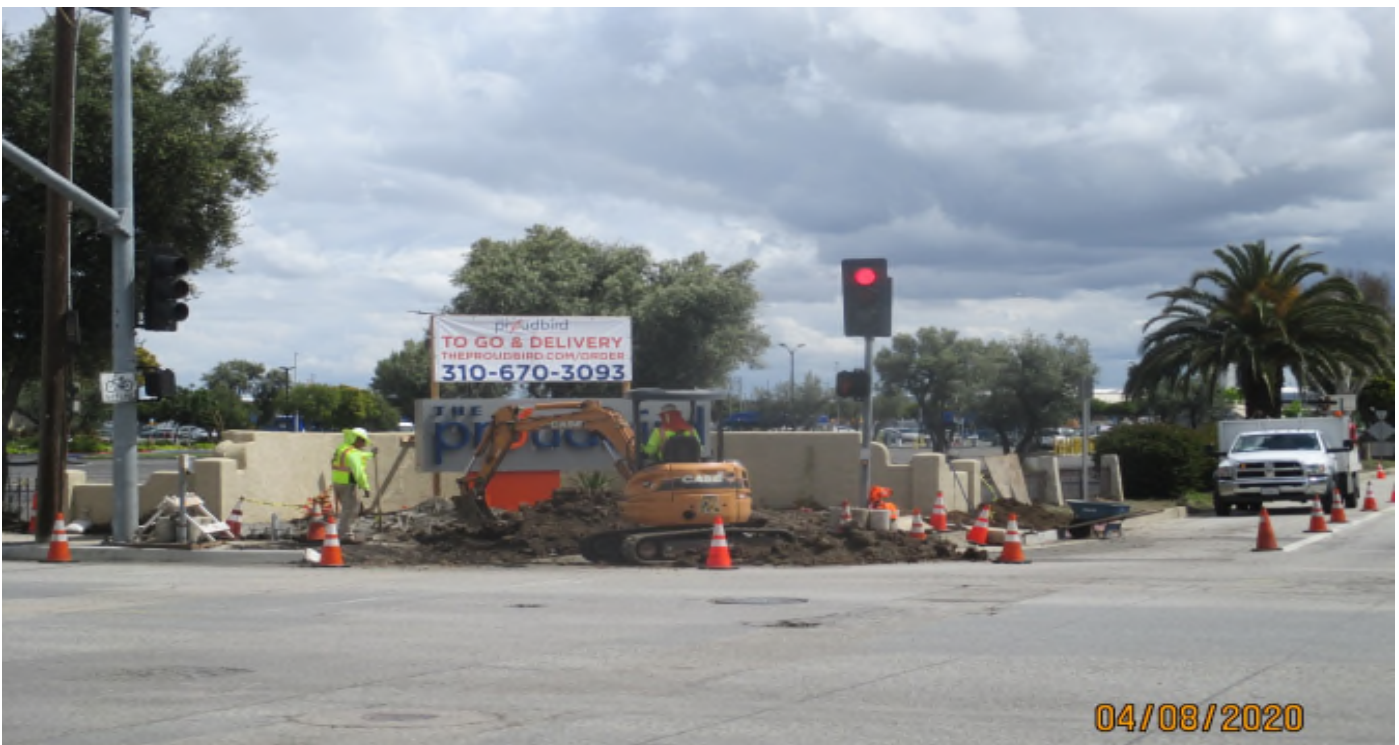
Aviation/Century – Traffic signal and street lighting conduit trenching on 111th and Aviation.
