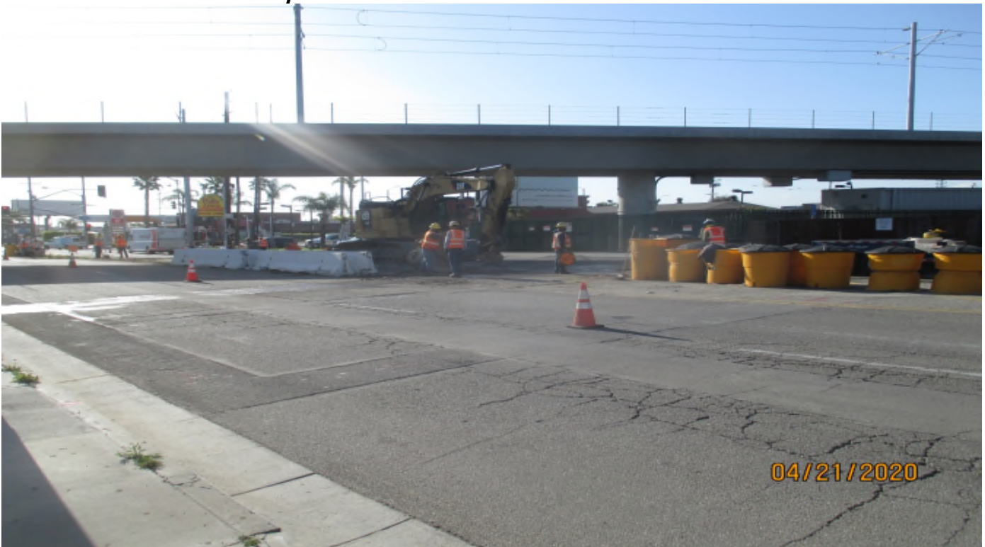
MANCHESTER STREET- Moving K rail and clean up to start the demo at Manchester.
