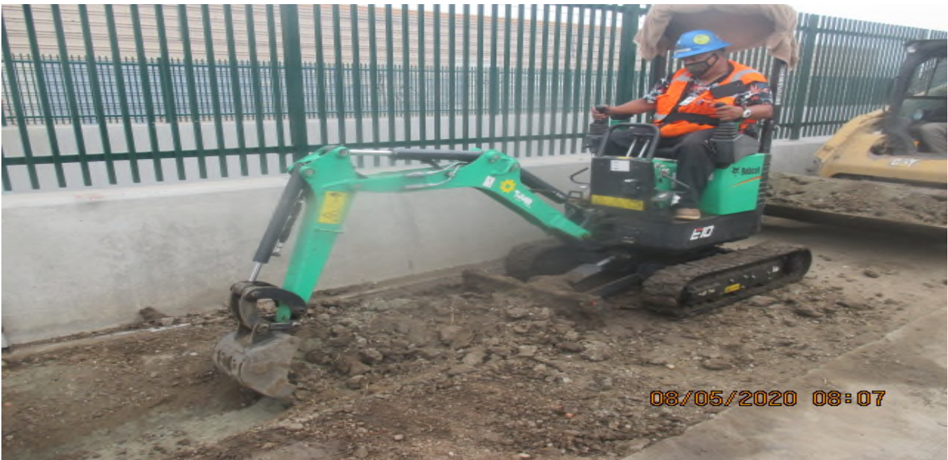
UG3 – Continue excavating for the culvert drainage system along the northbound barrier wall at Victoria Yard. 5/8/20
