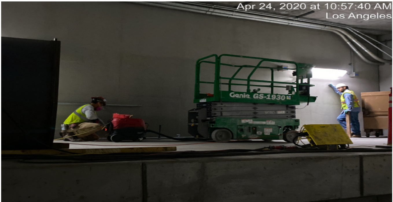
UG4 – WSCC in UG4 NB #4 track STA 371+64, repair work on emergency walkway foundations.
