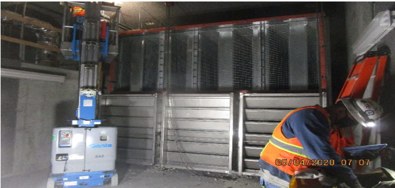
MLK STATION – Continue hardware support installation to TFD-7-322 in the North Tunnel Vent Plenum C – 140 of the concourse level.
