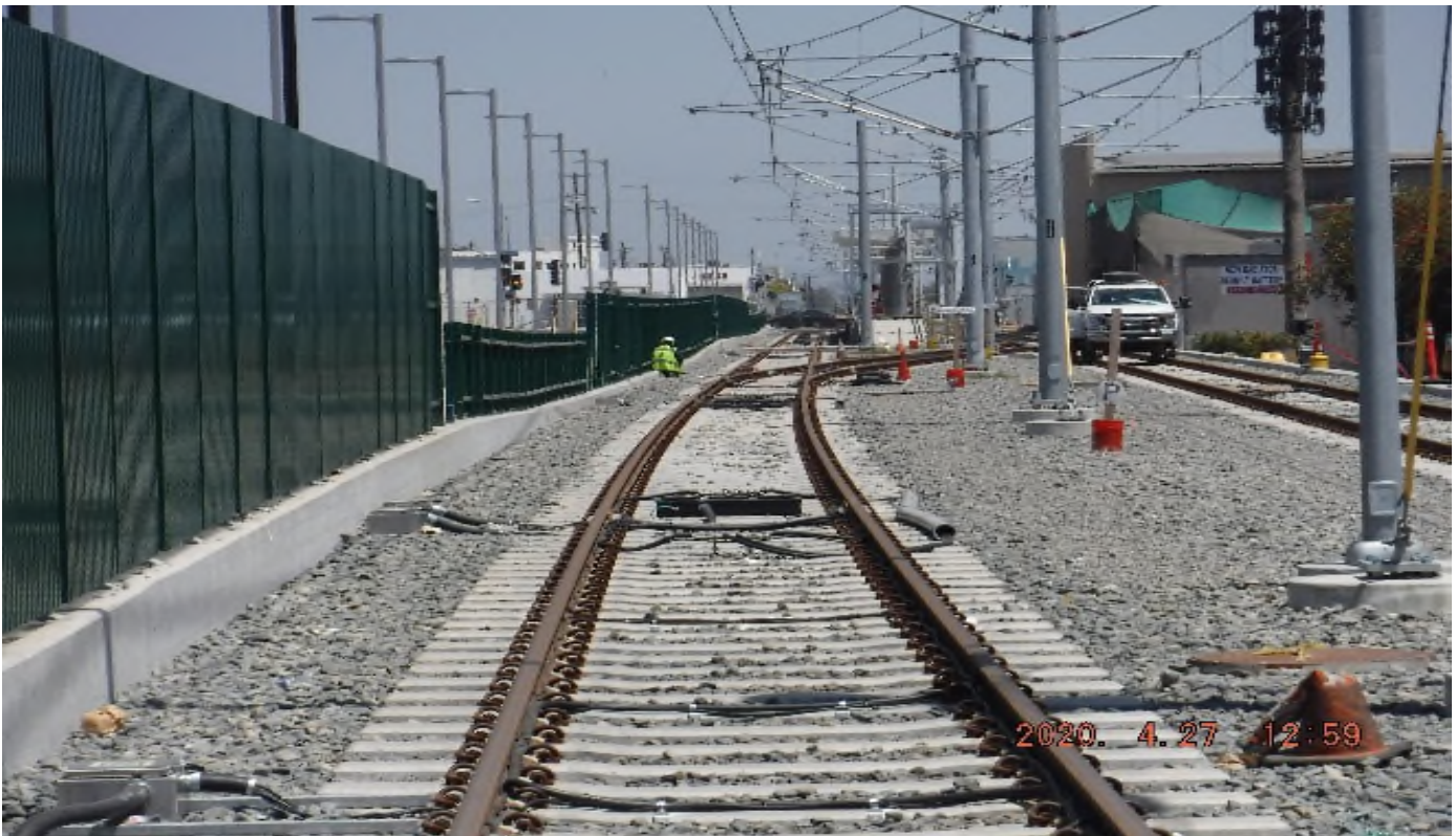
Florence/High St. - STA 257+30 TK#3/SB looking north – TC (system) work between High St (behind camera) and West Blvd.
