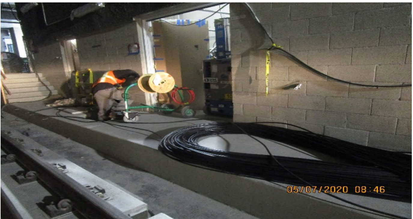
Crenshaw/Vernon - Vernon Concourse, Elevator 3 & 4 continued terminating control wiring (19 conductor #18) EM lighting & fans
