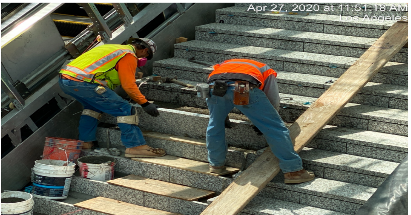
LEIMERT PARK STATION – Continue granite thread and riser installation at the main stair case landing of the plaza level.
