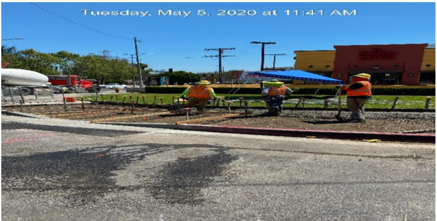
LEIMERT PARK STATION – Placing forms and concrete for new ADA ramp installation on the southeast corner of Vernon Ave and Crenshaw Blvd.
