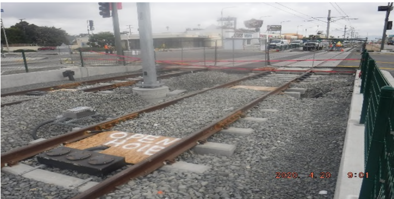
57th STREET-STA 329+40 TK#4,NB looking north – track status , track structure disturbance after weekend work NCR-B-089 (57th St) – PUNCH LIST
