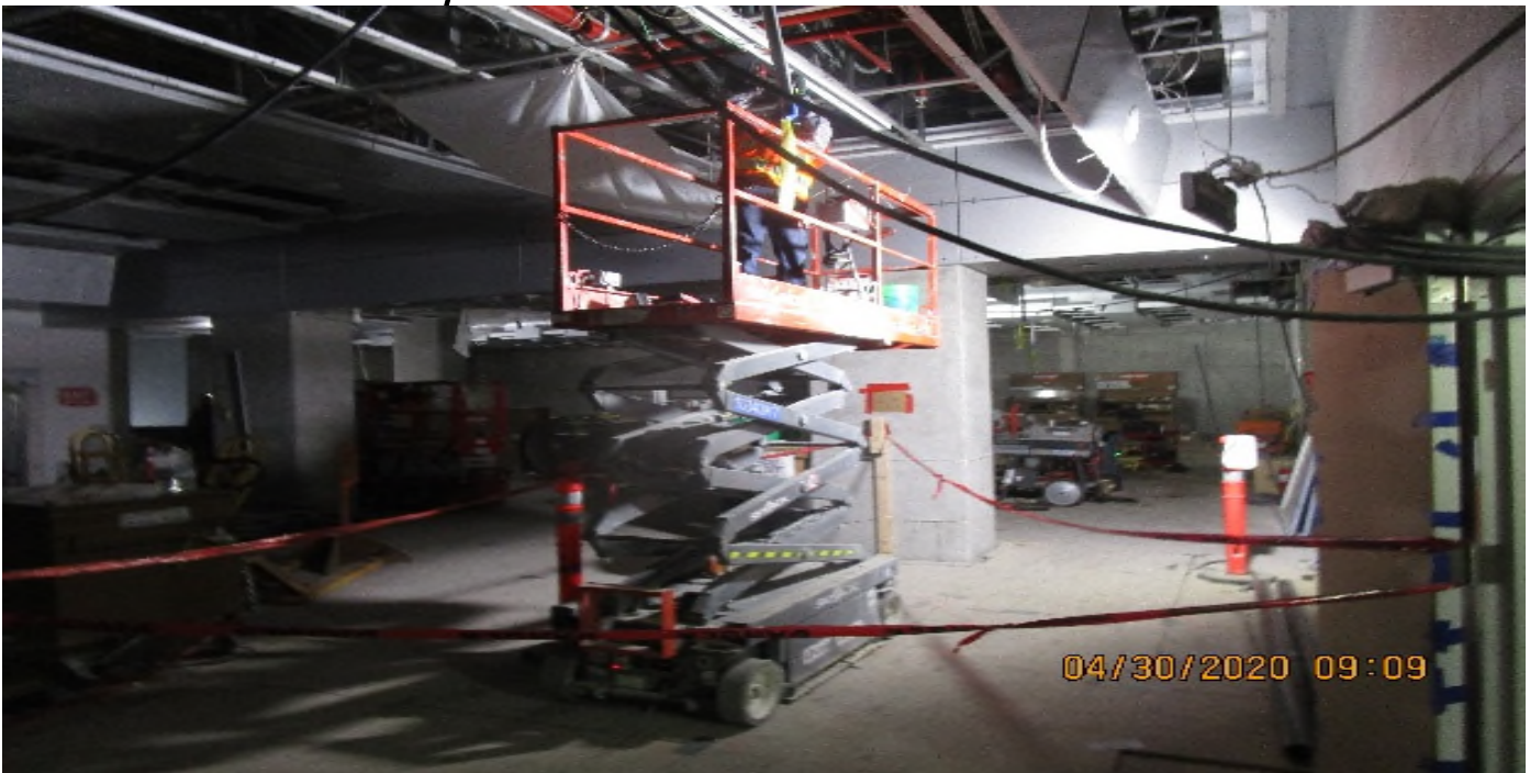
LEIMERT PARK STATION – Continue installing ceiling light fixtures at the concourse level.
