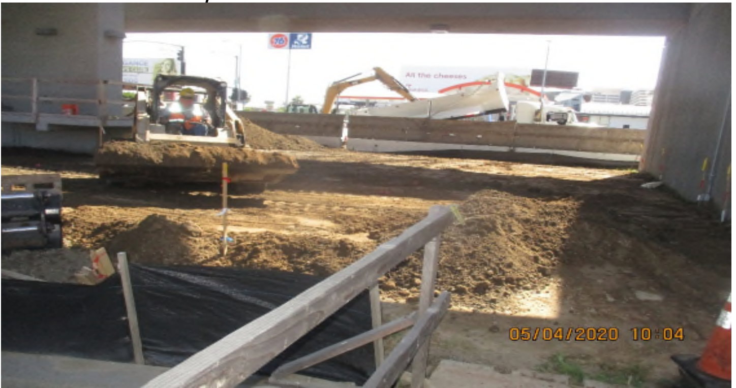
AVIATION/CENTURY - WSCC import soil and make grade at S/W COR of Aviation and Century.
