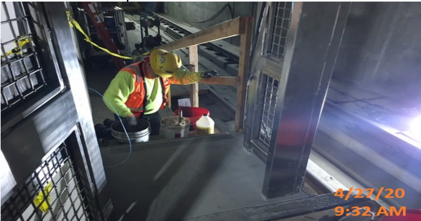
EXPO STATION – Surfacing and patching northbound stair landing on the south end of the platform level.
