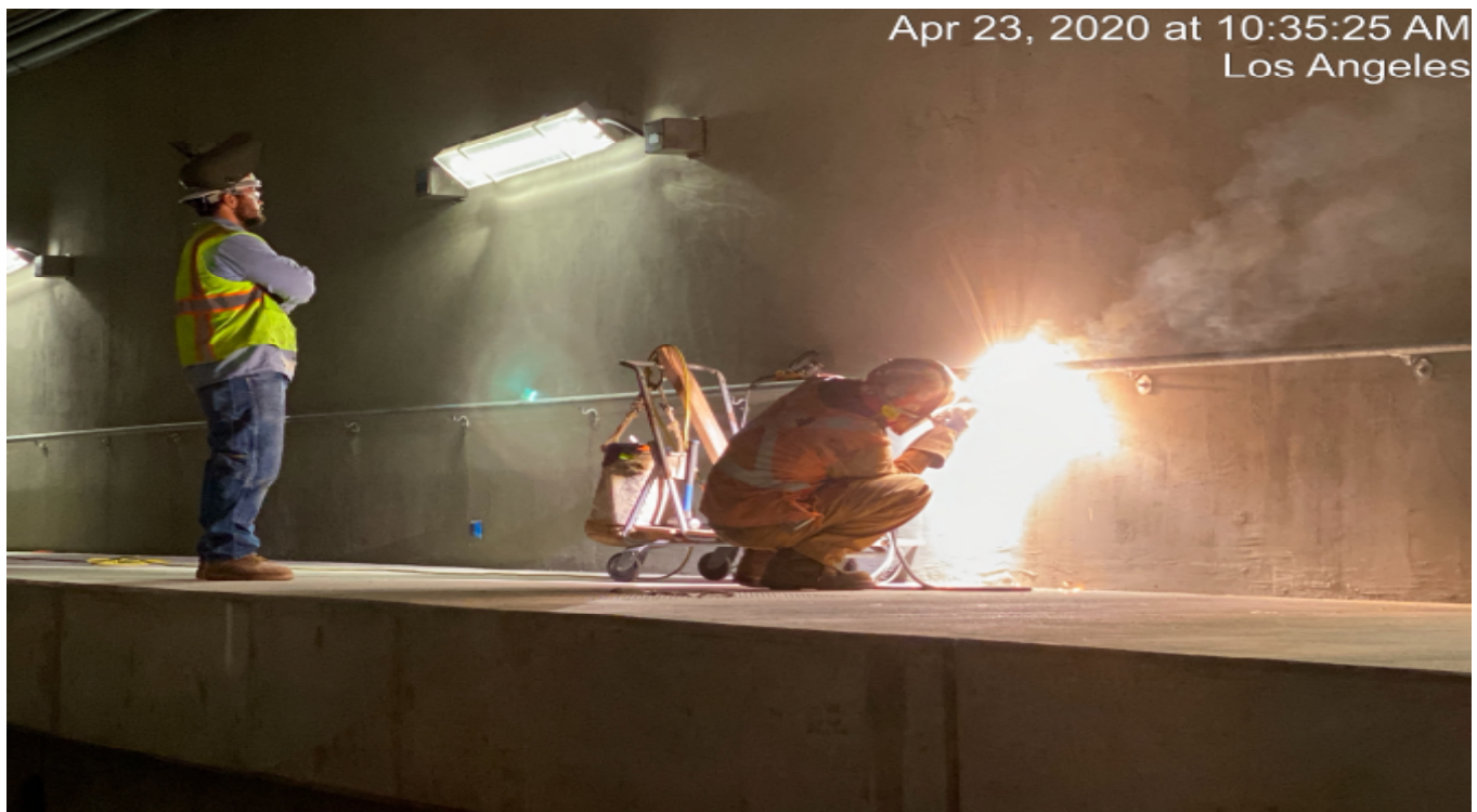
UG4 – Continue handrail installation for the emergency walkways along the northbound tunnel near the south portal entrance.
