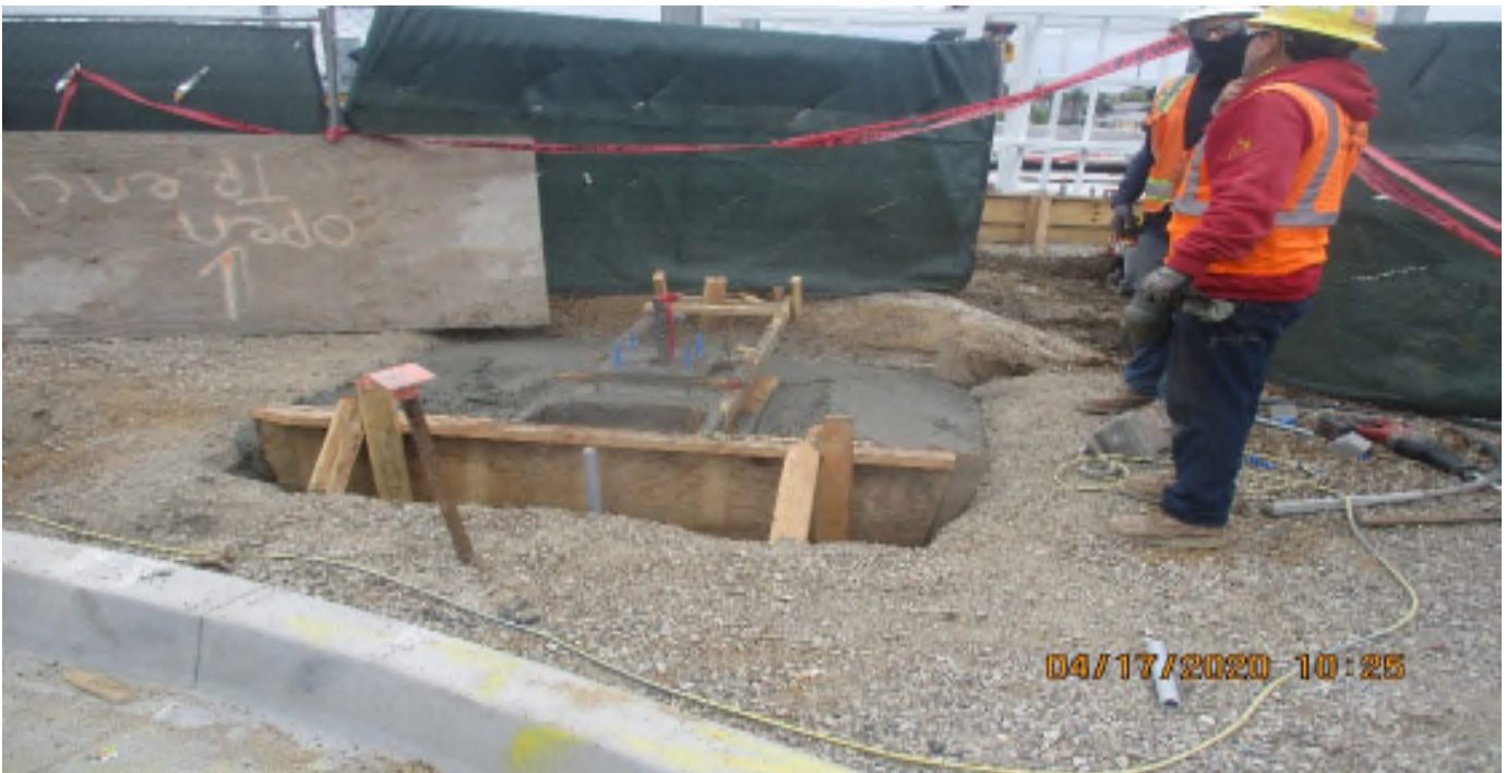
Florence/Brea – WSCC Placed concrete for pylons at W/B Florence at La Brea Station.
