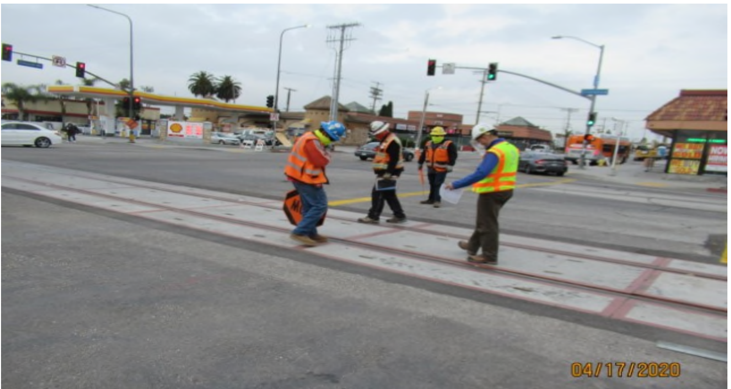
Crenshaw / Slauson – Slauson Ave grade crossing STA 323+88, Metro & WSCC inspectors verifying rail gouges on NB #4 track (looking northeast)
