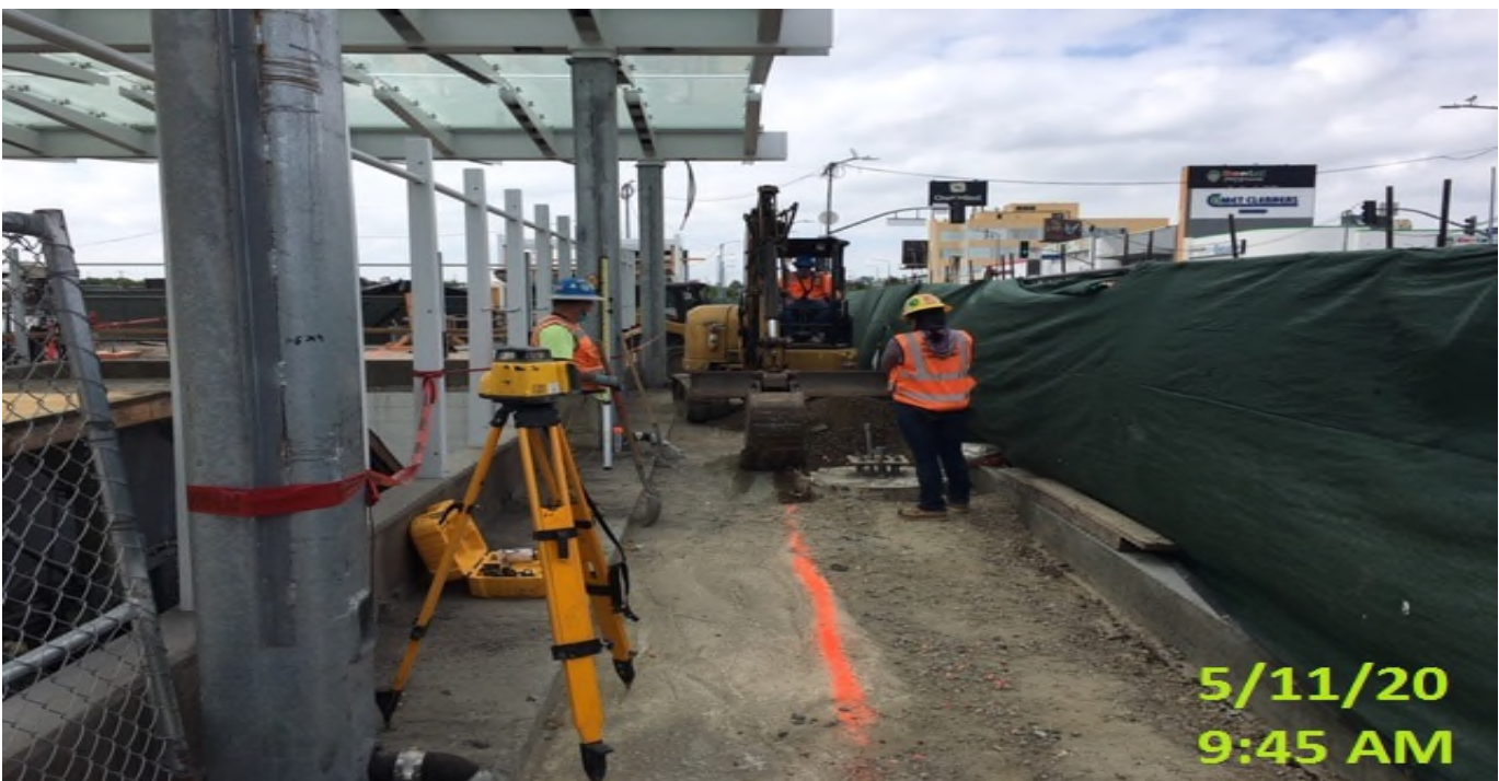
EXPO STATION – Continue trenching for conduit duct bank installation at the southwest corner of the plaza level.
