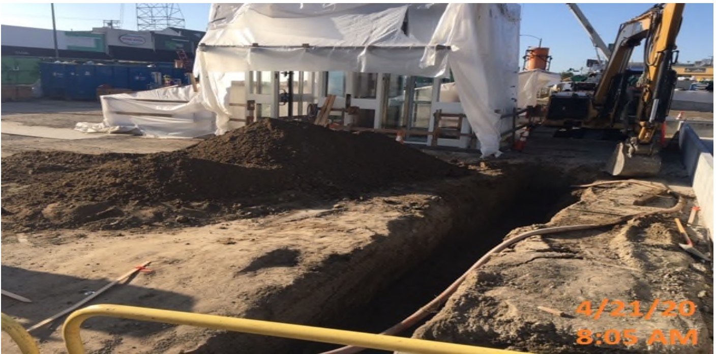
MLK STATION – Excavating for new 12” HDPE drainage pipe adjacent to Elevators 1&2 at the plaza level.
