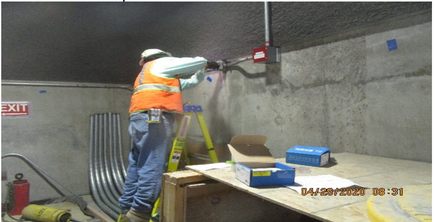
Crenshaw/Vernon - Vernon Emergency ventilation shaft equipment access (S) C107 begin installing horn strobe devices, ID & label
