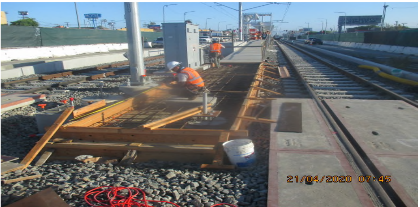
Hyde Park Station – Began formwork and rebar installation for the south end entrance ramp of the platform. 4/21/20
