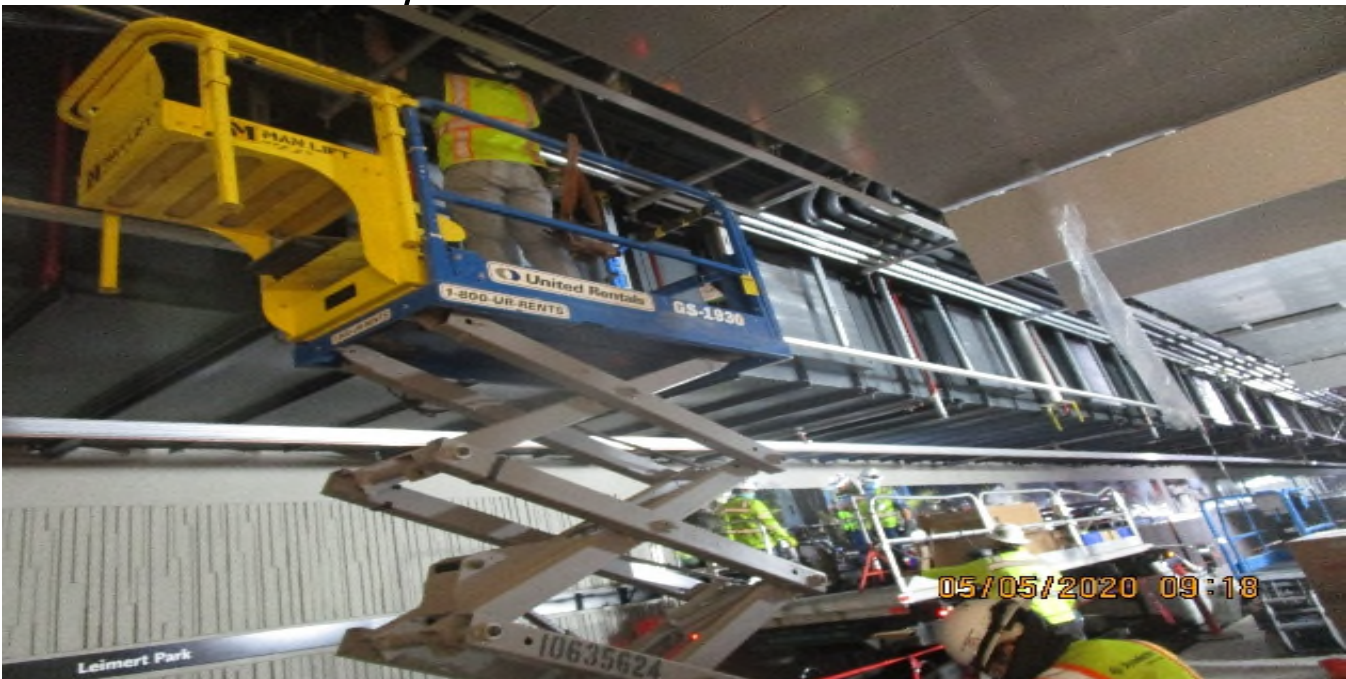
Crenshaw/Vernon - Vernon North Platform, Continued overhead bonding Radiax GRC (5) 2" GRC with #2 7-strand bare copper grounds
