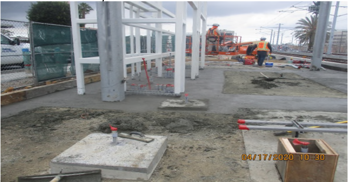
Florence/Brea – WSCC Placed concrete for platform at South ticket pavilion at La Brea Station.
