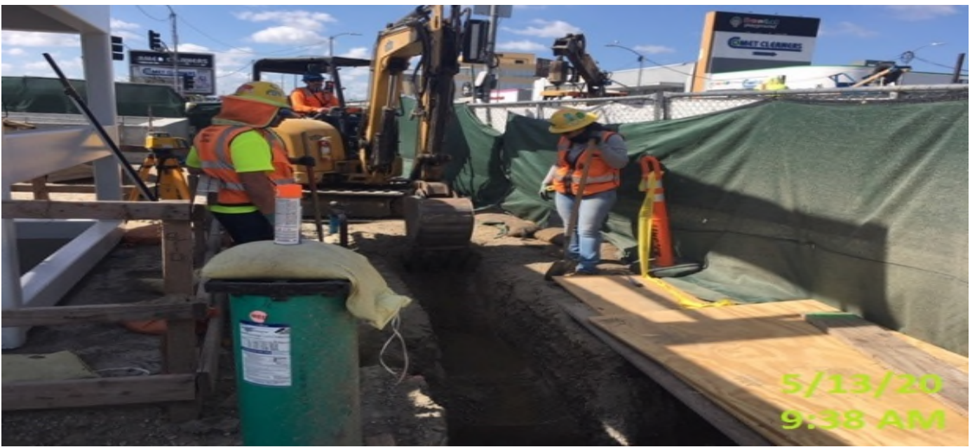
EXPO STATION – Continue trenching for conduit duct bank installation at the southwest corner of the plaza level.
