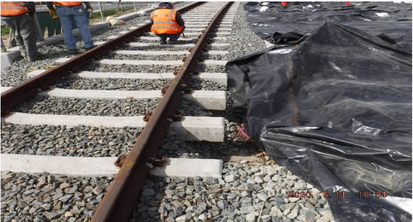
Florence/Brea - STA 206+00 TK#4,NB looking south – track geometry measurement south of La Brea Station – missing track ballast left shoulder
