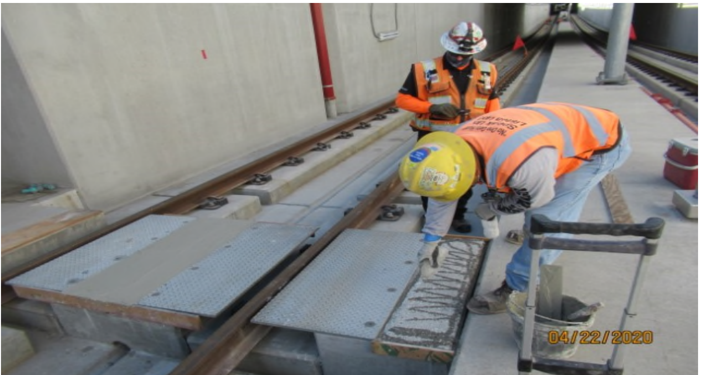
UG1 – WSCC repair work on emergency walkway crossing in UG1 SB #3 track STA 49+73
