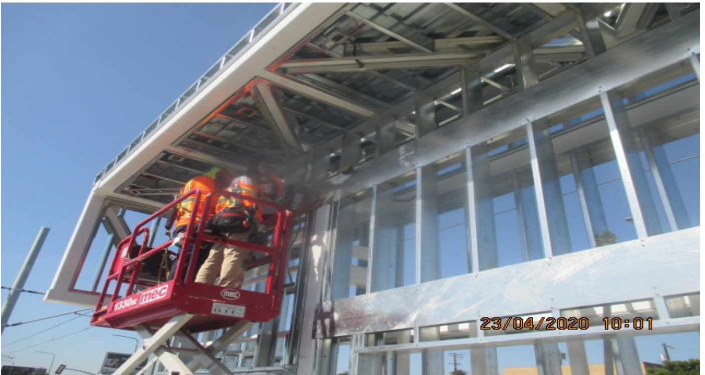
Hyde Park Station –Installing utility and lighting on both the north and south end canopy structures. 4/23/20
