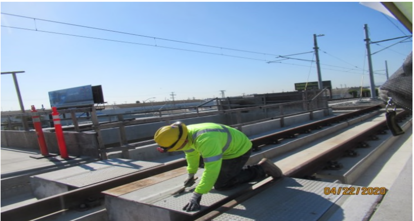
AVIATION/CENTURY- WSCC finalizing elevations on grout for emergency walkway crossing on SB #3 track STA 66+16 Century, Aviation bridge (looking southeast) Rework
