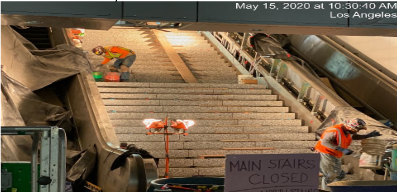
LEIMERT PARK STATION – Continue granite thread and riser installation at the concourse stair case landing.
