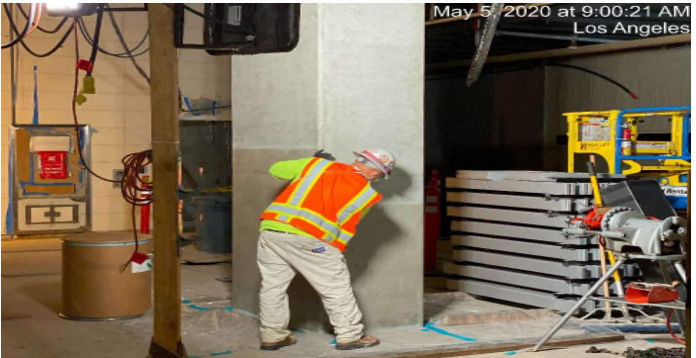
LEIMERT PARK STATION – Applying anti-graffiti finish coat to all the columns at the platform level.
