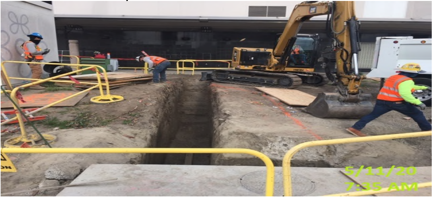
MLK STATION – Continue excavating for 12” HDPE drainage pipe system at the northwest section of the plaza level.
