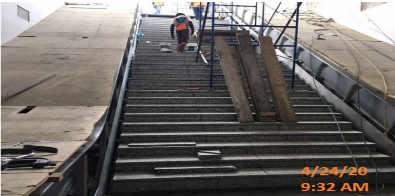
EXPO STATION – Continue granite stair landing section installation at the main entrance staircase of the plaza level.
