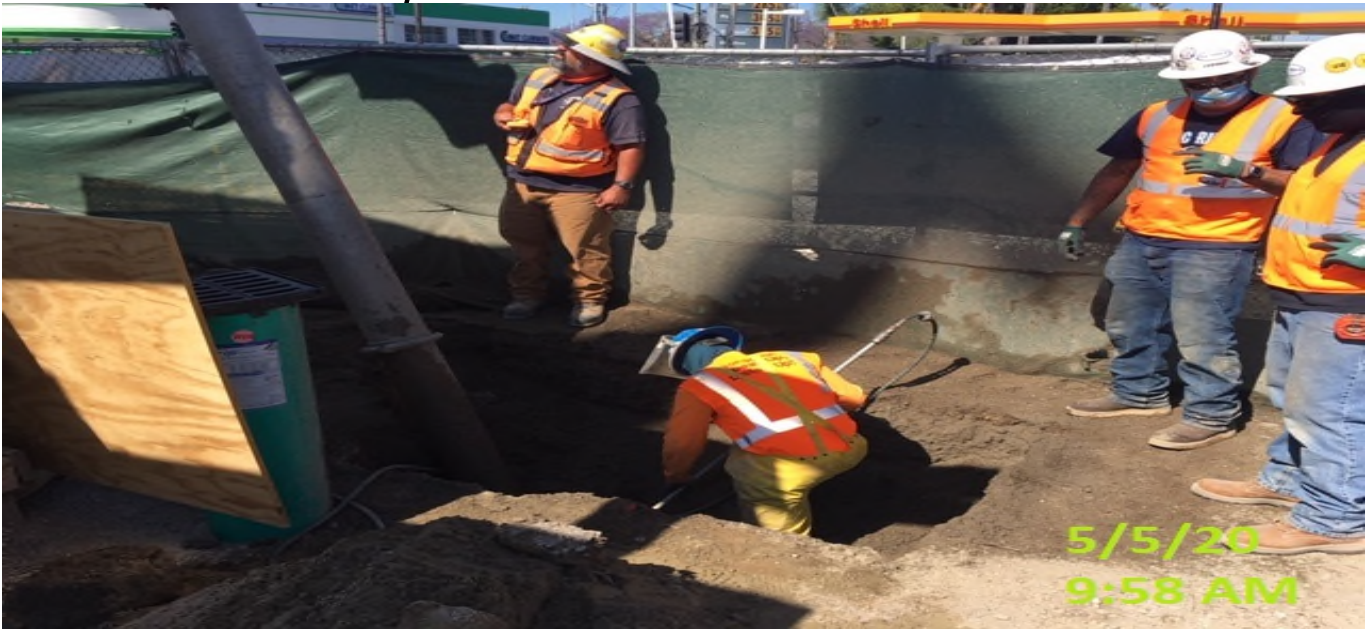
EXPO STATION – Potholing for conduit duct bank installation at the southwest corner of the plaza level.
