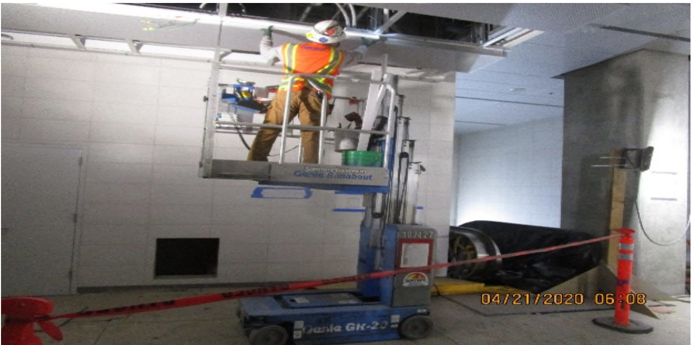
LEIMERT PARK STATION – Continue installing ceiling light fixtures at the concourse level.
