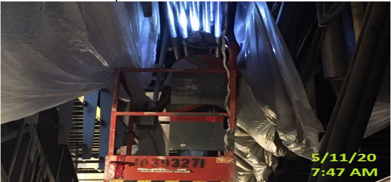
MLK STATION – Continue preparing for primer application to the ceiling conduits at the platform level.
