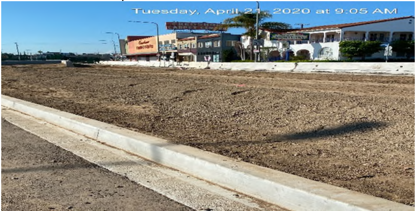
LEIMERT PARK STATION – Continue backfilling/grading the center guideway median island for drainage on Crenshaw Blvd between 48th St and Vernon Ave.
