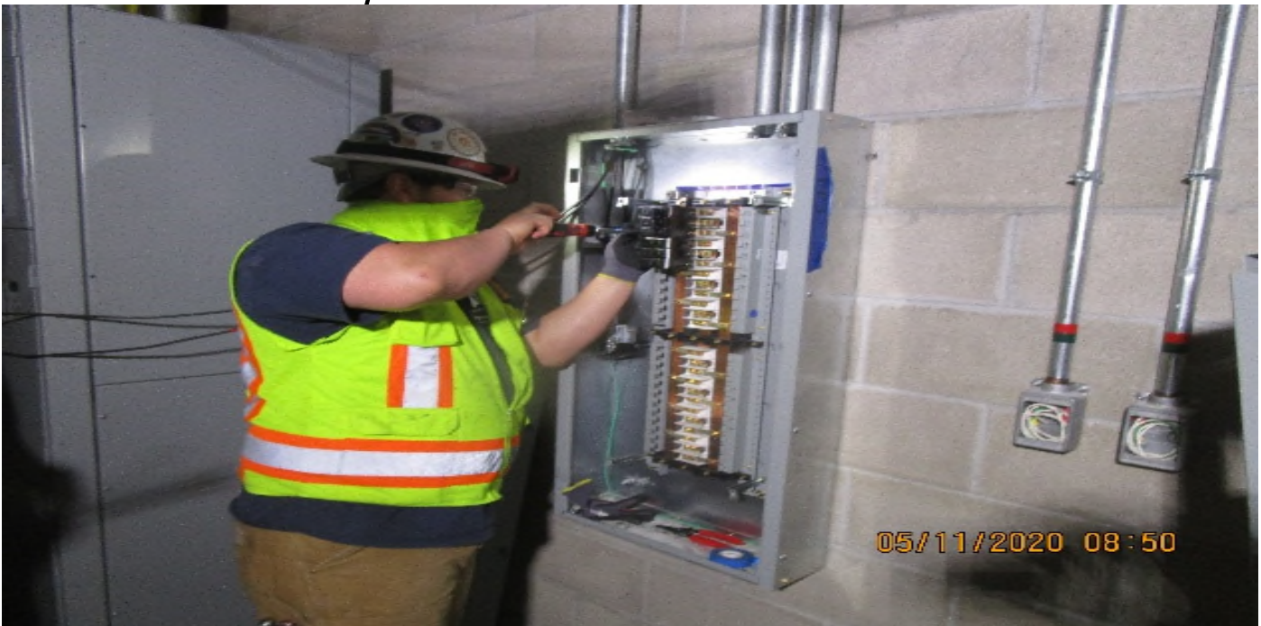
Crenshaw/Vernon - Vernon Concourse, TC&C Room C112. Begin dressing & terminating #10 grounds at distribution panel PP3/S
