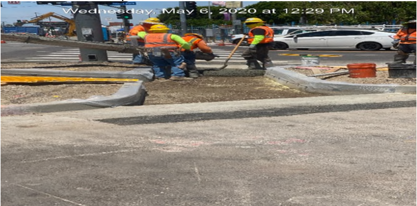
LEIMERT PARK STATION – Placing concrete for new walkway and dome installation on the southeast corner of Vernon Ave and Crenshaw Blvd.
