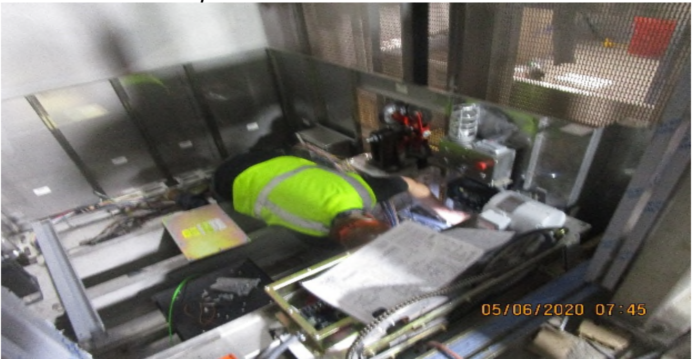
Crenshaw/Vernon - Vernon Concourse, Elevator 3 & 4 continued terminating control wiring (19 conductor #18) EM lighting & fans
