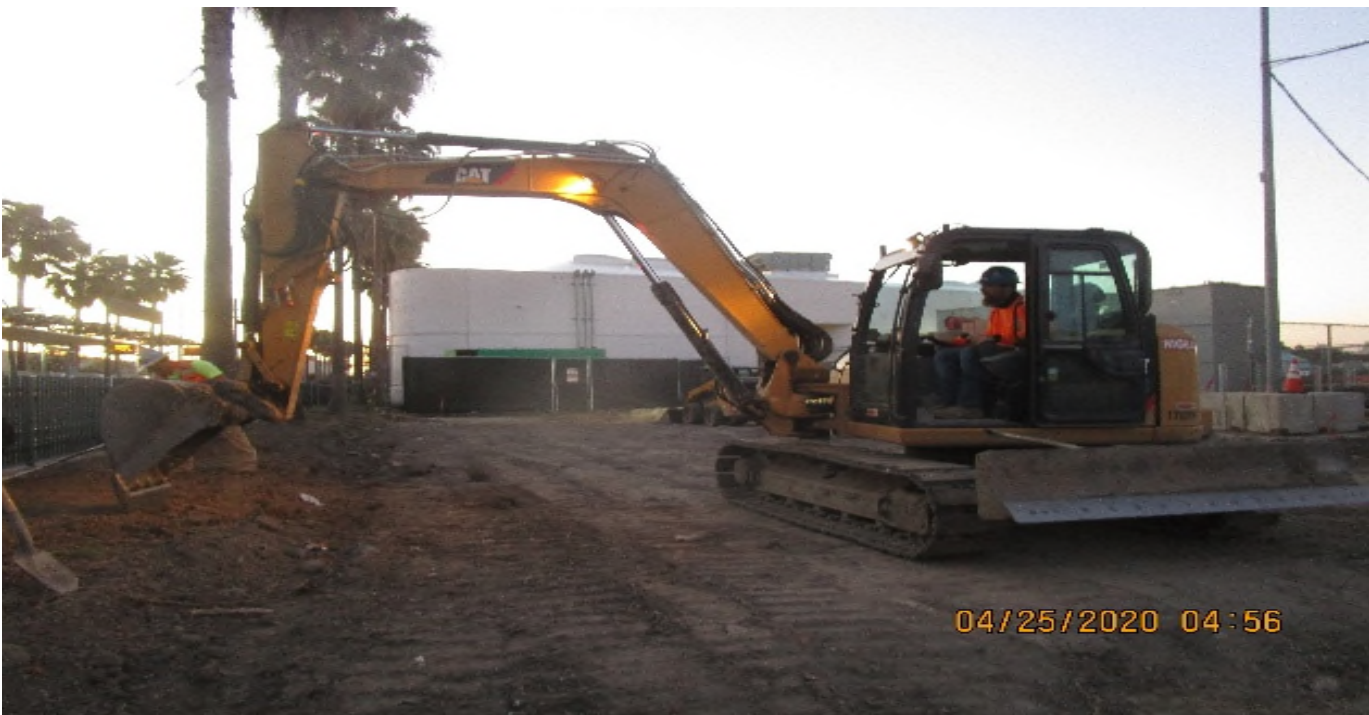
EXPO STATION – Grading for upcoming treatment swale installation on the east end of the plaza level.
