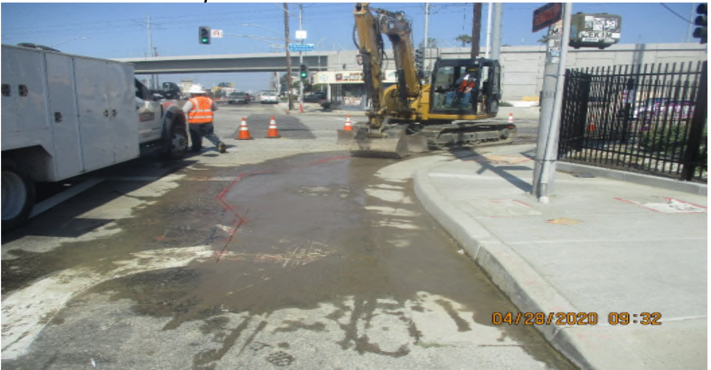
Manchester Bridge – WSCC Saw cut and remove street at N/E corner of Manchester and Florence.
