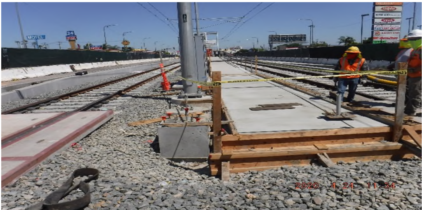
Crenshaw / Slauson - STA 317+00 TK#3/SB looking north – form removal around pedestrian landing south end Slauson Station
