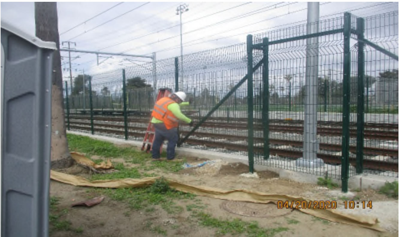
Florence/High St. - ACE Fence Placed fence panels at Florence west of High Street.
