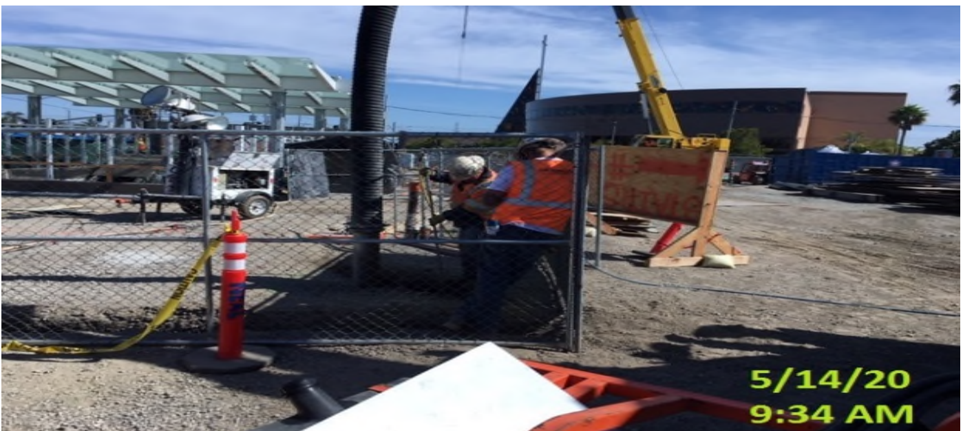
EXPO STATION – Continue potholing for upcoming tree well installation throughout the plaza level.
