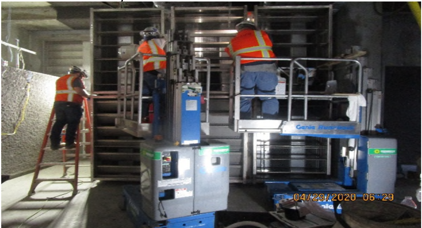
Crenshaw/MLK - MLK, Tunnel vent plenum southwest C103, continued rough in actuators & limit switches at TFD-7-121.
