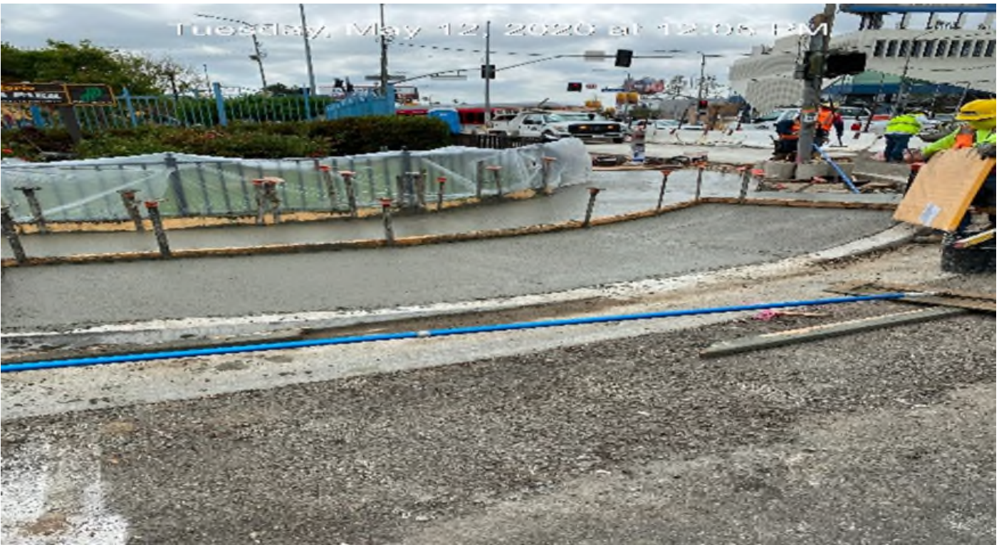
LEIMERT PARK STATION – Built formwork and placed concrete at the southeast corner of 43rd Pl and Crenshaw Blvd.
