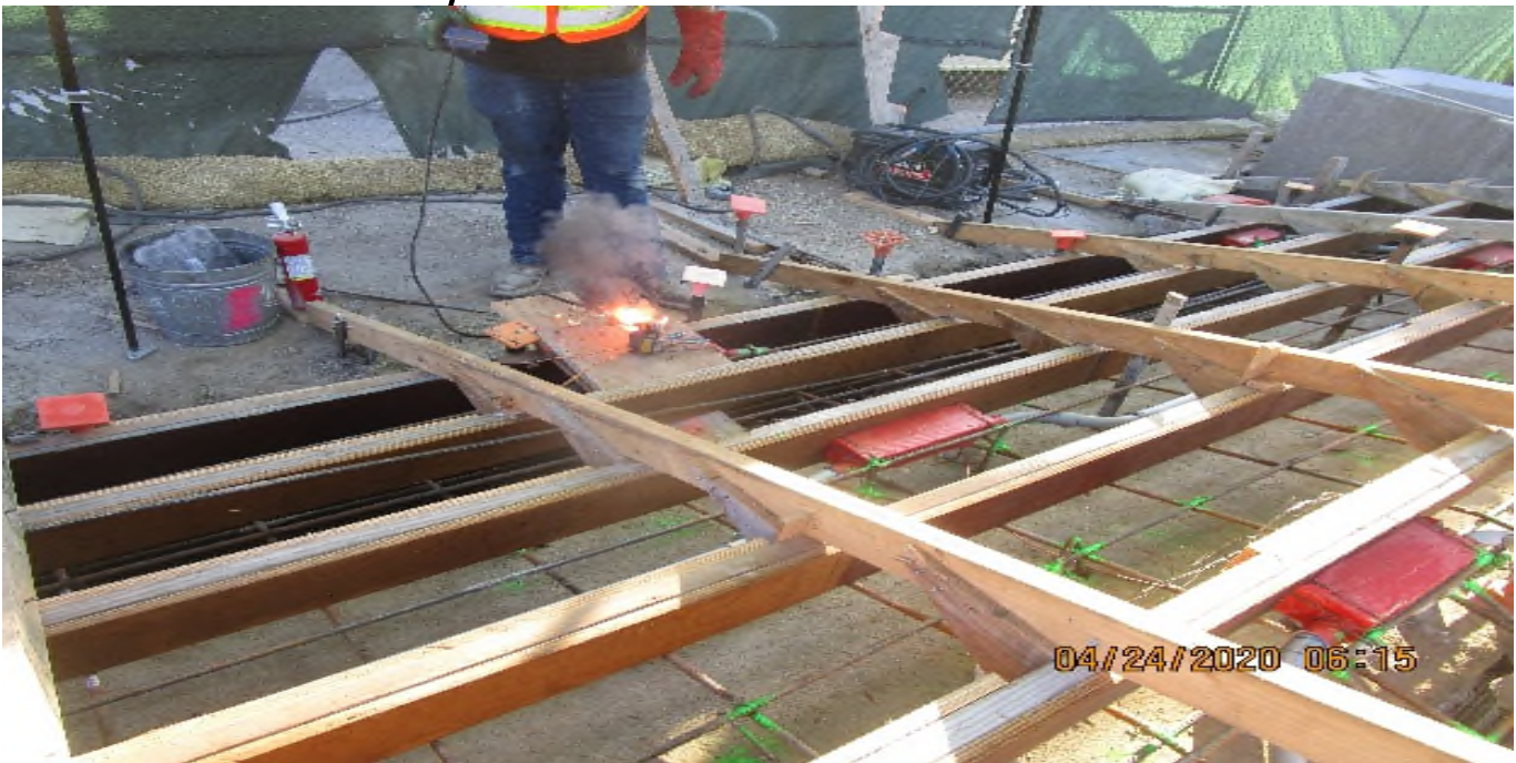
LEIMERT PARK STATION – Continue embedded and ramp lighting fixture installation for the planter stair risers on the northwest section of the plaza level.
