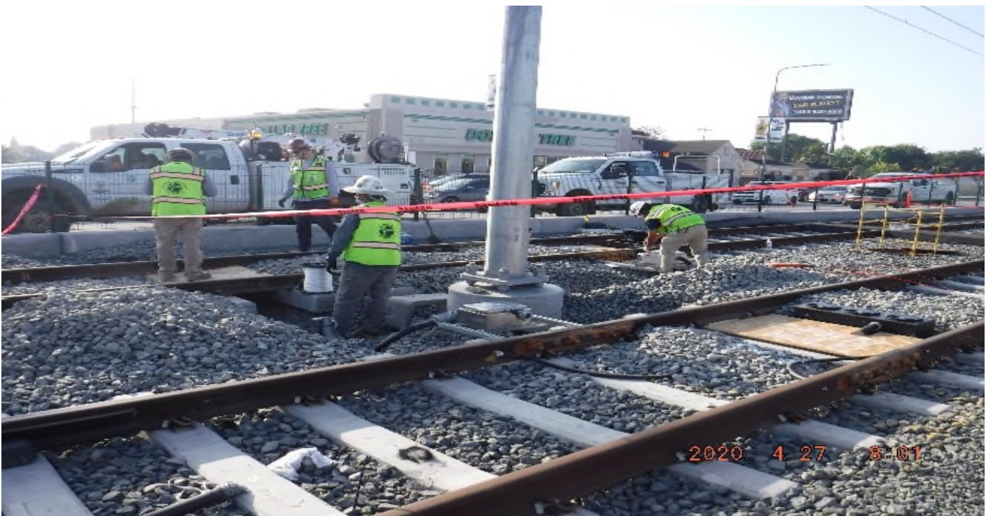
57 th Street - STA 330+00 TK#3/SB looking south (east) – system work with track structure disturbance south of 57th St around/next to OCS #1258 and MH-S099 – PUNCH LIST
