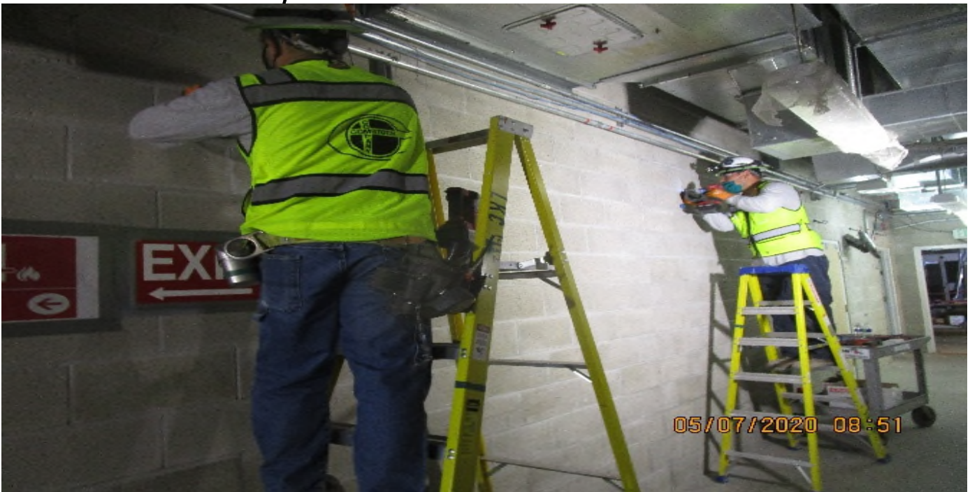
Crenshaw/Vernon - Vernon, Vestibule 3, C133 begin installing Radiax cable support brackets 5' On center East & West CMU walls
