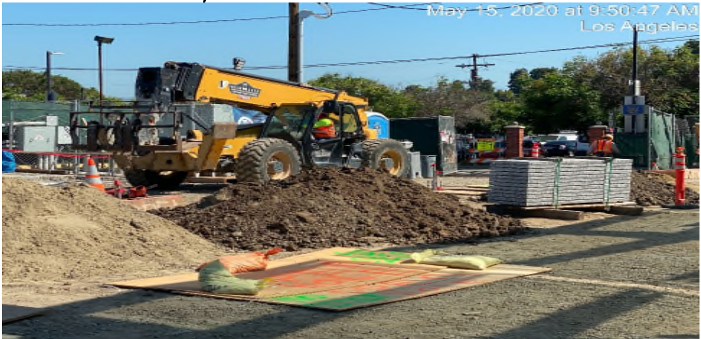
LEIMERT PARK STATION – Continue excavating for palm tree installation at the plaza.
