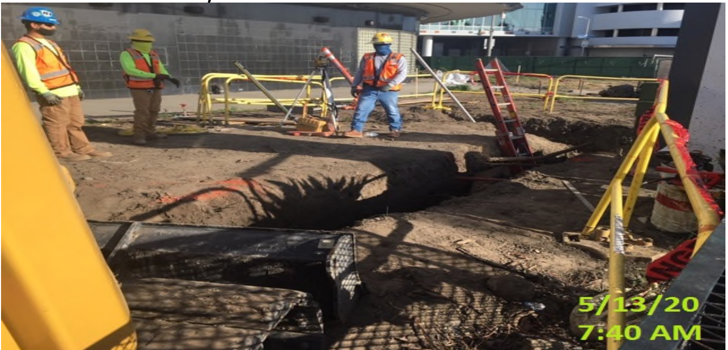
MLK STATION – Continue laying out 12” HDPE drainage pipe system at the northwest section of the plaza level.
