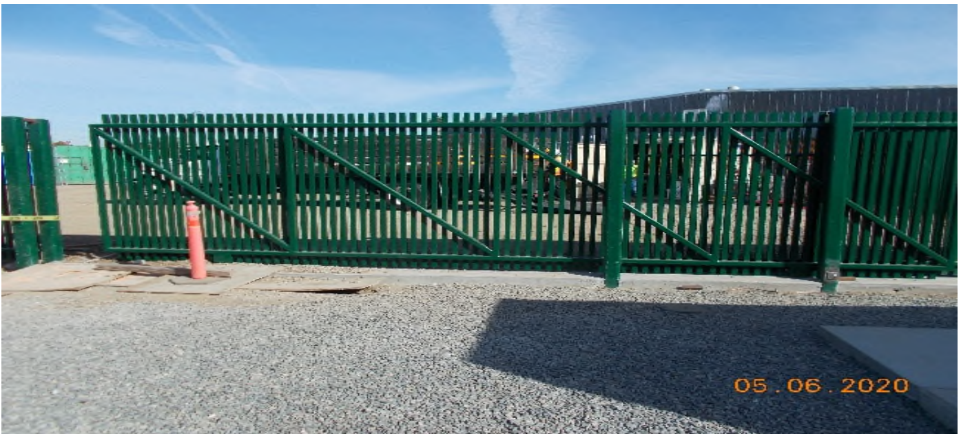
UG3 – Delivered and installed sliding gate for the entrance of the Auxiliary Power Bungalow at Victoria Yard.
