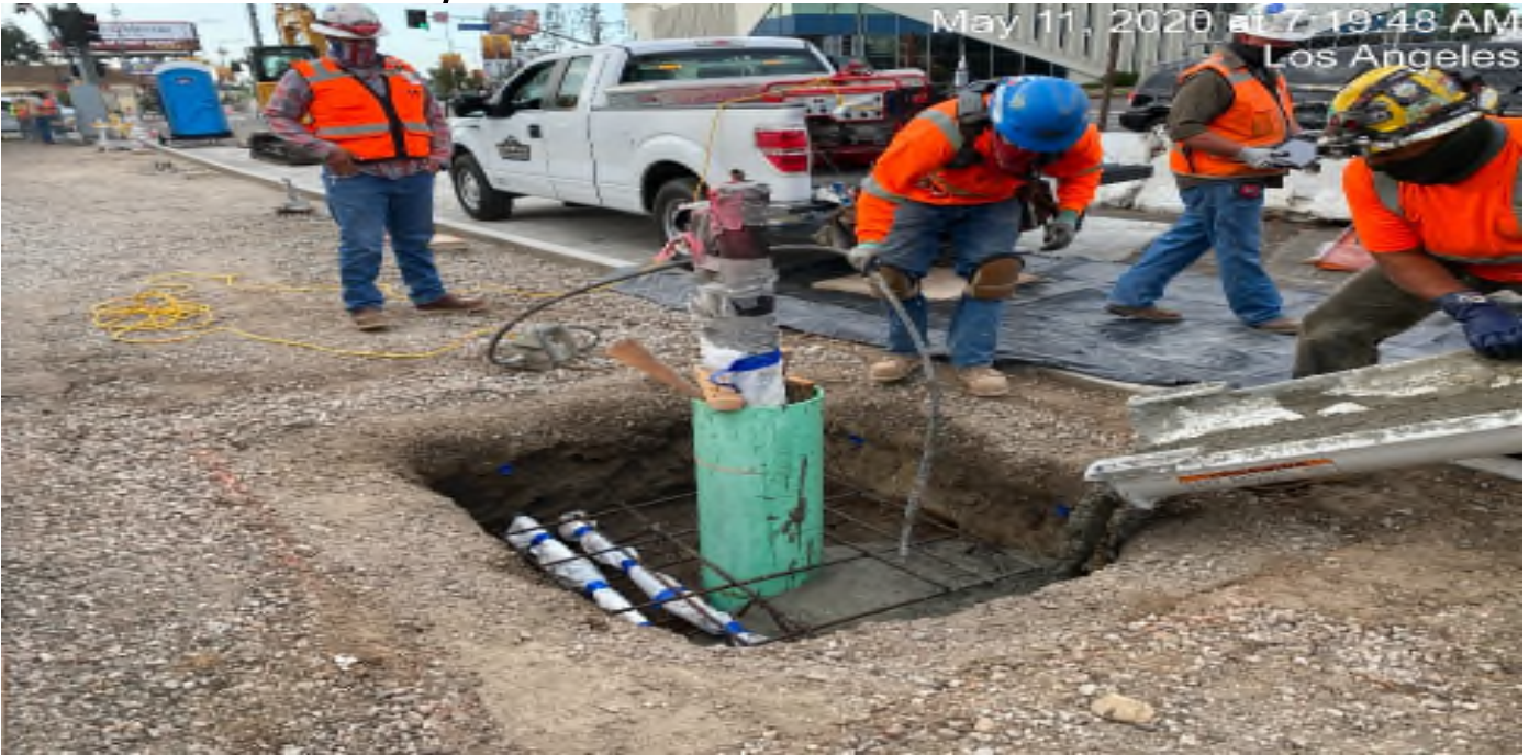
LEIMERT PARK STATION – Placing concrete for the plumping vent stack foundation on the southeast corner of 43rd Pl and Crenshaw Blvd.
