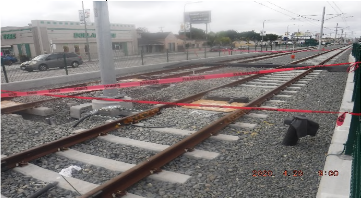
57th STREET- STA 330+00 TK#3 , SB looking south – system work with track structure disturbance south of 57th St around,next to OCS #1258 as of 4.20.2020 – PUNCH LIST
