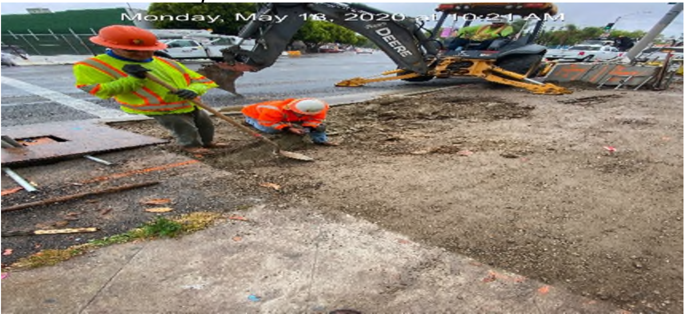
LEIMERT PARK STATION – Excavating for street light conduit installation on Crenshaw Blvd between 43rd Pl and Homeland Dr.
