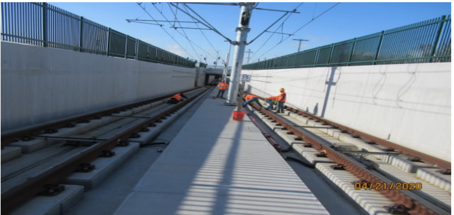
UG1 - WSCC crew in UG1 both NB & SB tracks, for install of epoxy on expansion joints (looking south) out of sequence work.
