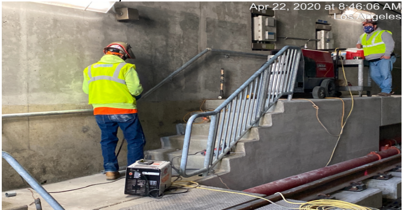
UG4 – Continue handrail installation for the emergency walkways along the southbound tunnel near the south portal entrance.
