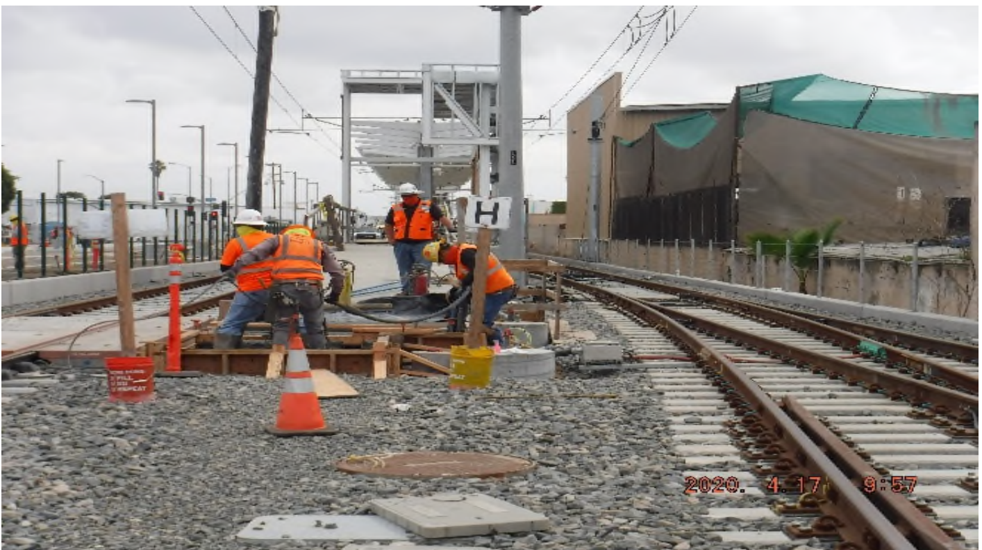
Florence/West – STA 262+75 TK#3/SB looking north – pour PCC for pedestrian landing south end of West Station Platform.
