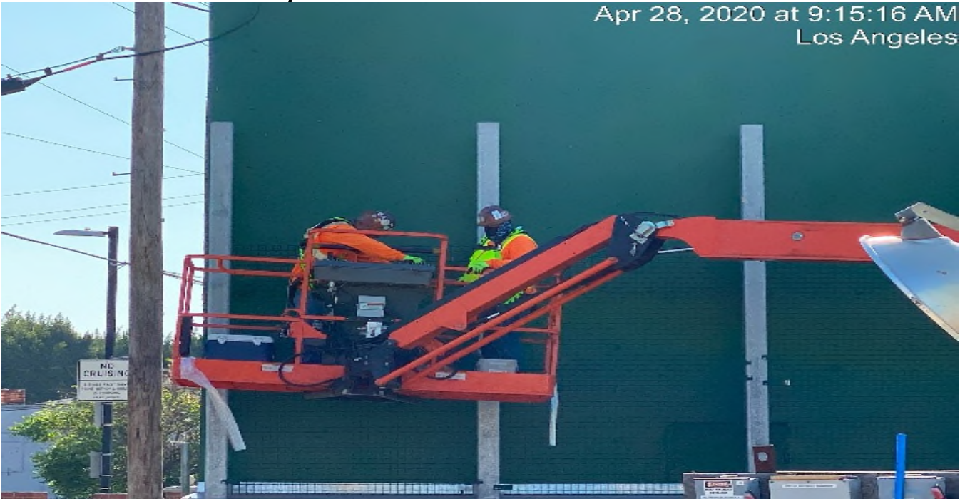
LEIMERT PARK STATION – Continue lattice installation for the green screen wall at the plaza level.
