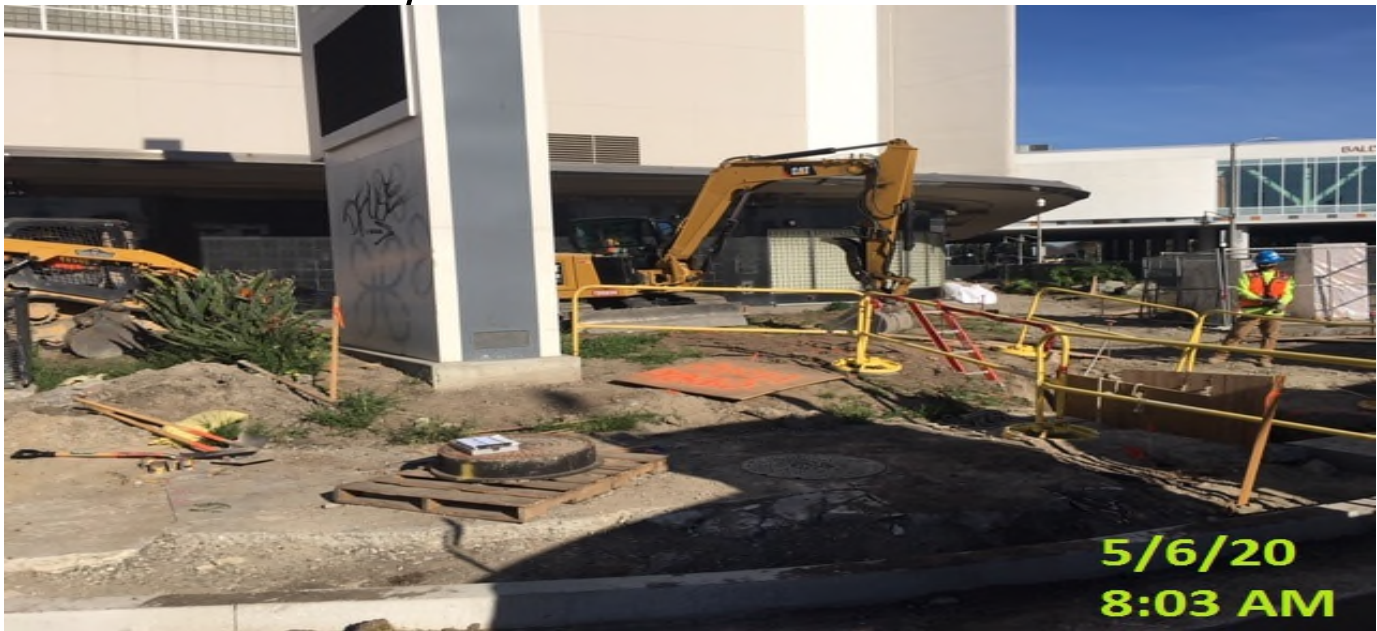
MLK STATION – Continue trenching for 12” HDPE drainage pipe system at the northern section of the plaza level.
