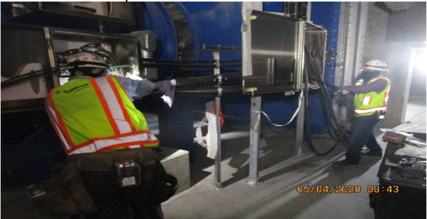
MLK Concourse, Emergency fan room (S) C102 Begin pulling EVF-6-121 (6) 500 kcmils feeders & (9) 1/0's.
