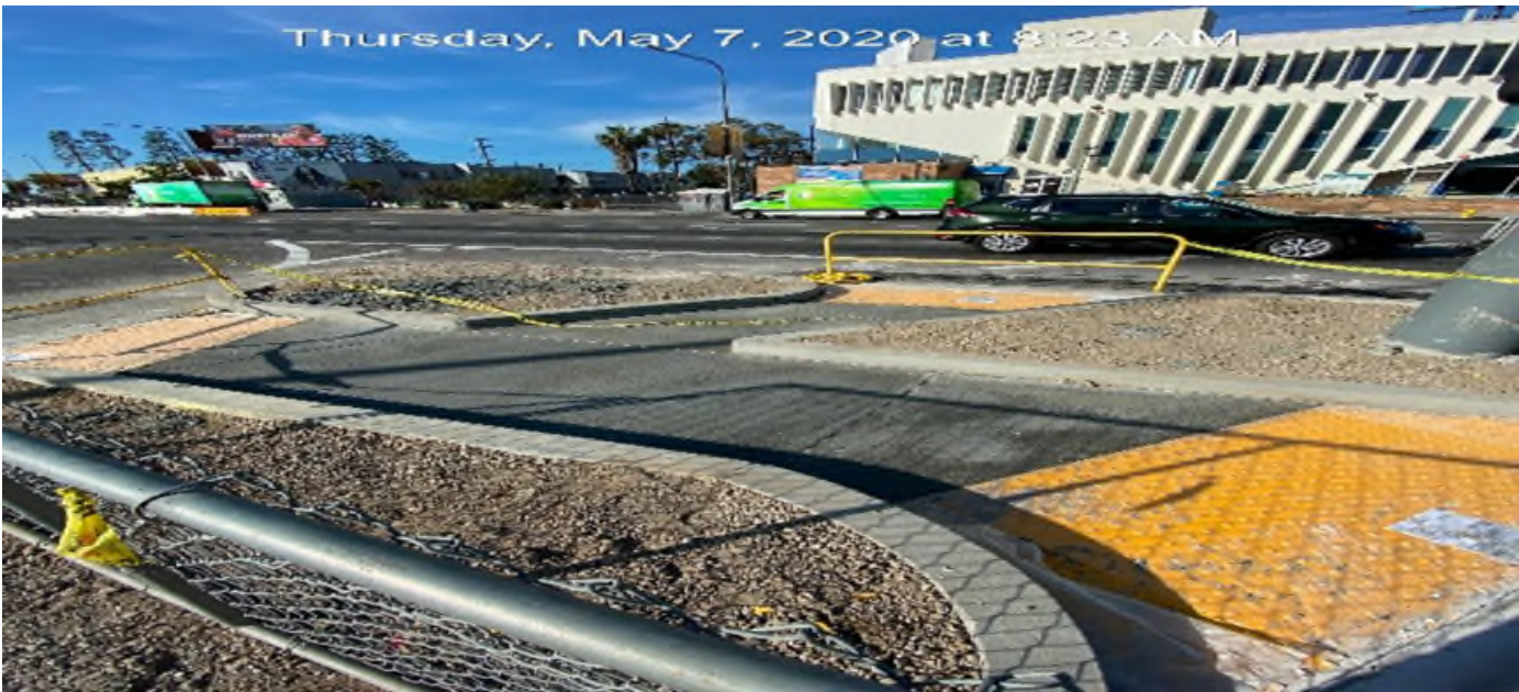
LEIMERT PARK STATION – Completed concrete placement of walkway and domes for the southeast corner of Vernon Ave and Crenshaw Blvd.
