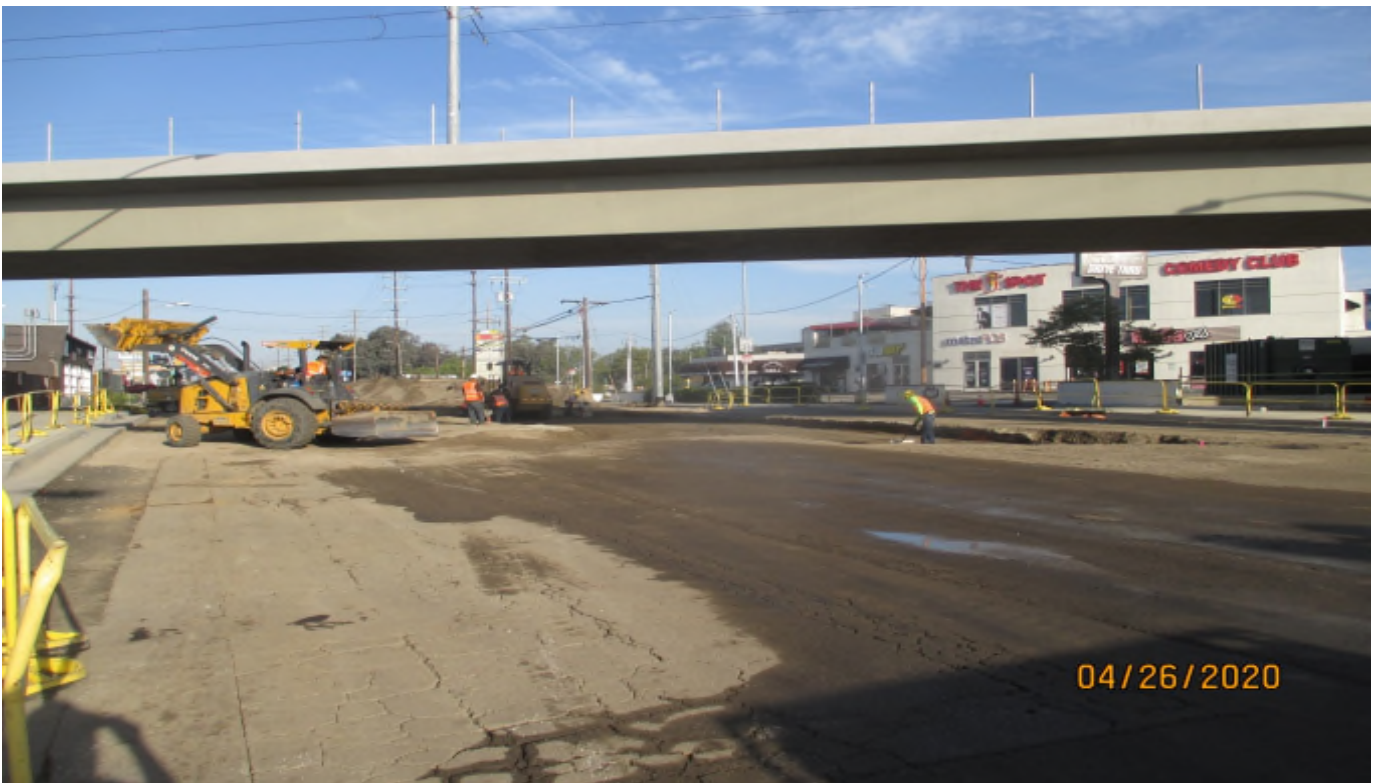
MANCHESTER STREET- Compaction of the base for the median and #1 WB lane on Manchester.
