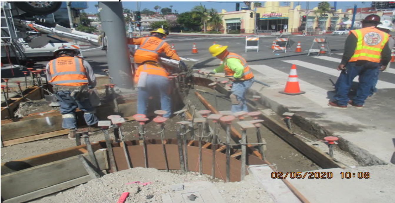
LEIMERT PARK STATION – Placing forms and concrete for new curb/gutter installation on the southeast corner island of Vernon Ave and Crenshaw Blvd. 5/2/20
