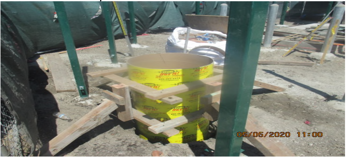
PARK MESA – Began sonotube formwork and rebar installation for light pole foundations at the northeast corner of TPSS#7 on 60th St & Crenshaw Blvd. 5/5/20
