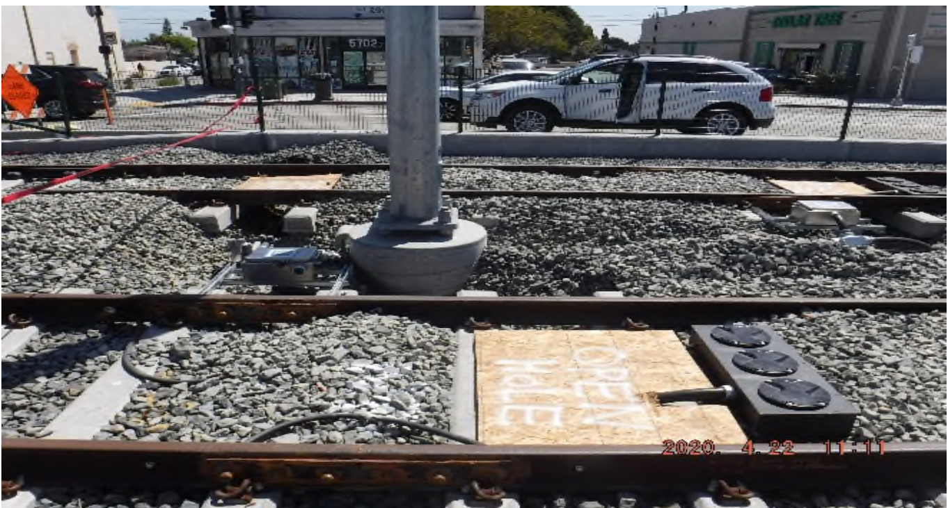
57th STREET- STA 329+75 TK#3,SB looking east – system work with track structure disturbance south of 57th St around,next to OCS #1258 as of 4.22.2020 – PUNCH LIST
