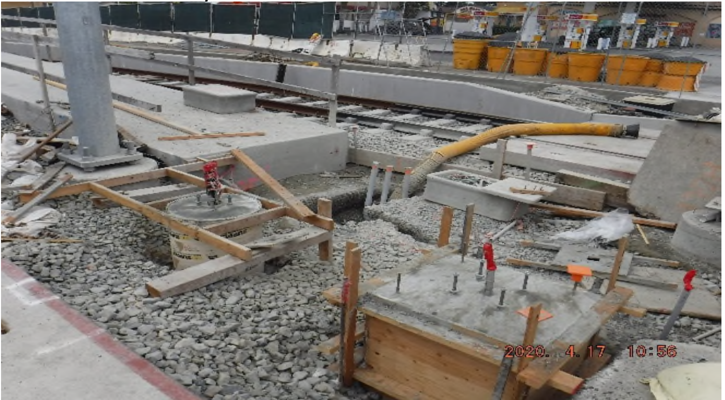
Crenshaw / Slauson - STA 323+00 TK#4/NB looking south – dirt spilled all over track ballast after pole foundation excavation north end Slauson Sta
