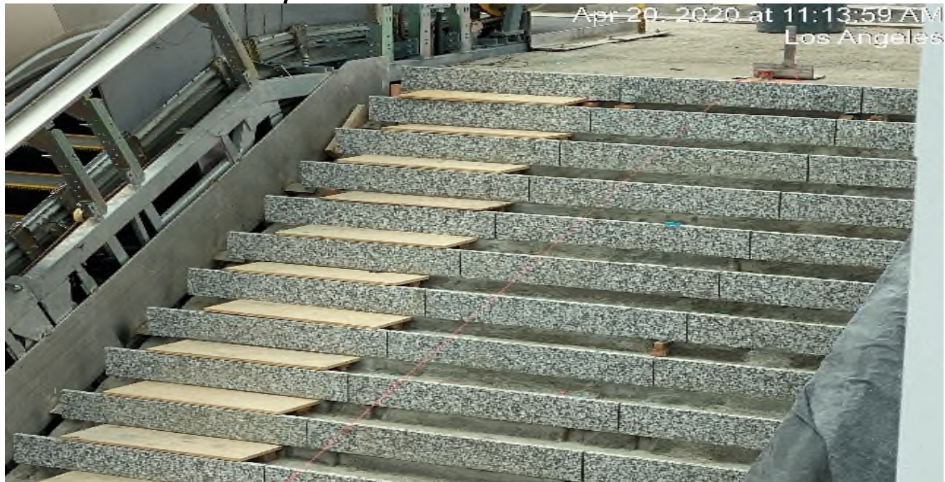
LEIMERT PARK STATION – Continue granite thread and riser installation at the main stair case landing of the plaza level.
