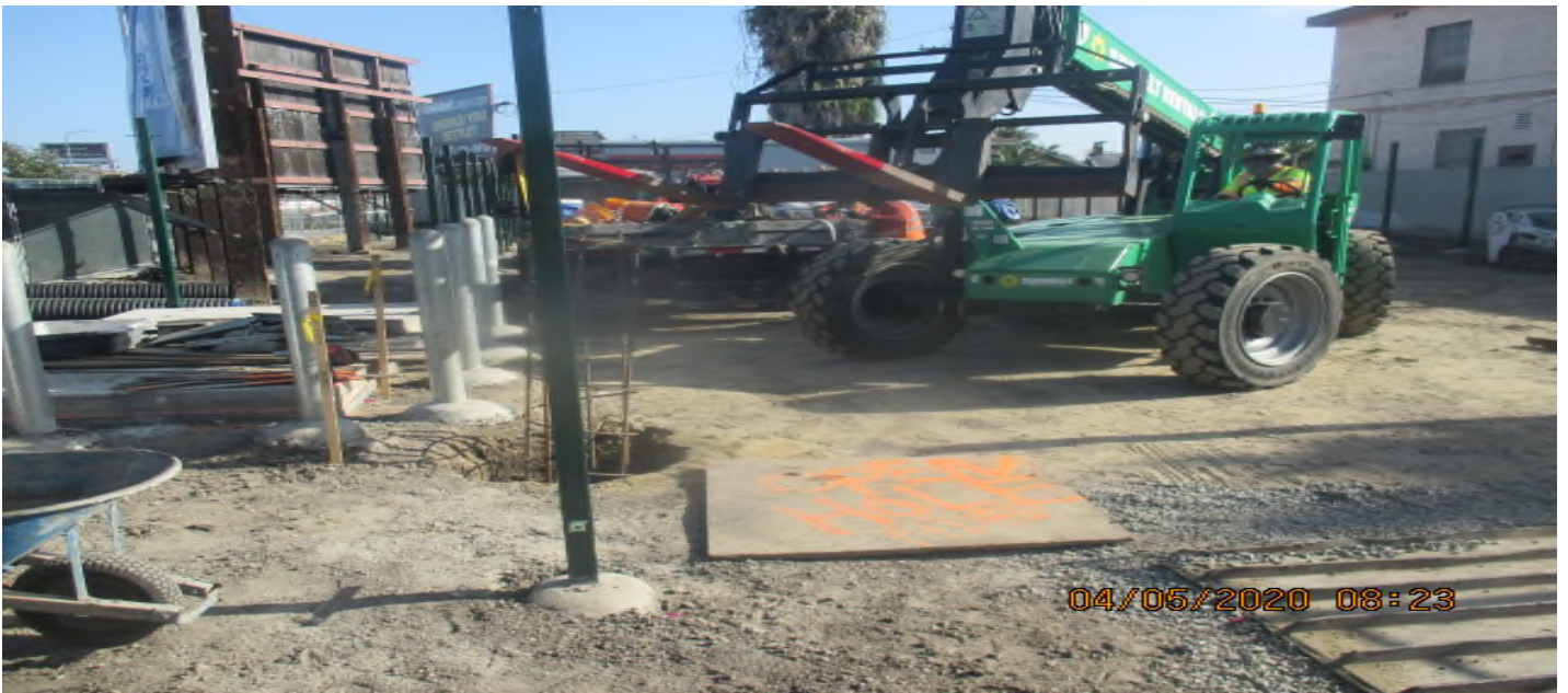
PARK MESA – Continue fence post installation around the perimeter of TPSS#7 on 60th St & Crenshaw Blvd. 5/4/20
