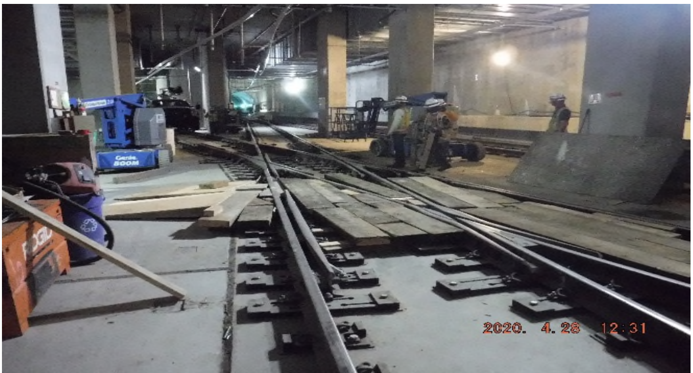
UG-4- Continue pulling wire for the emergency lighting at the south end portal entrance.
