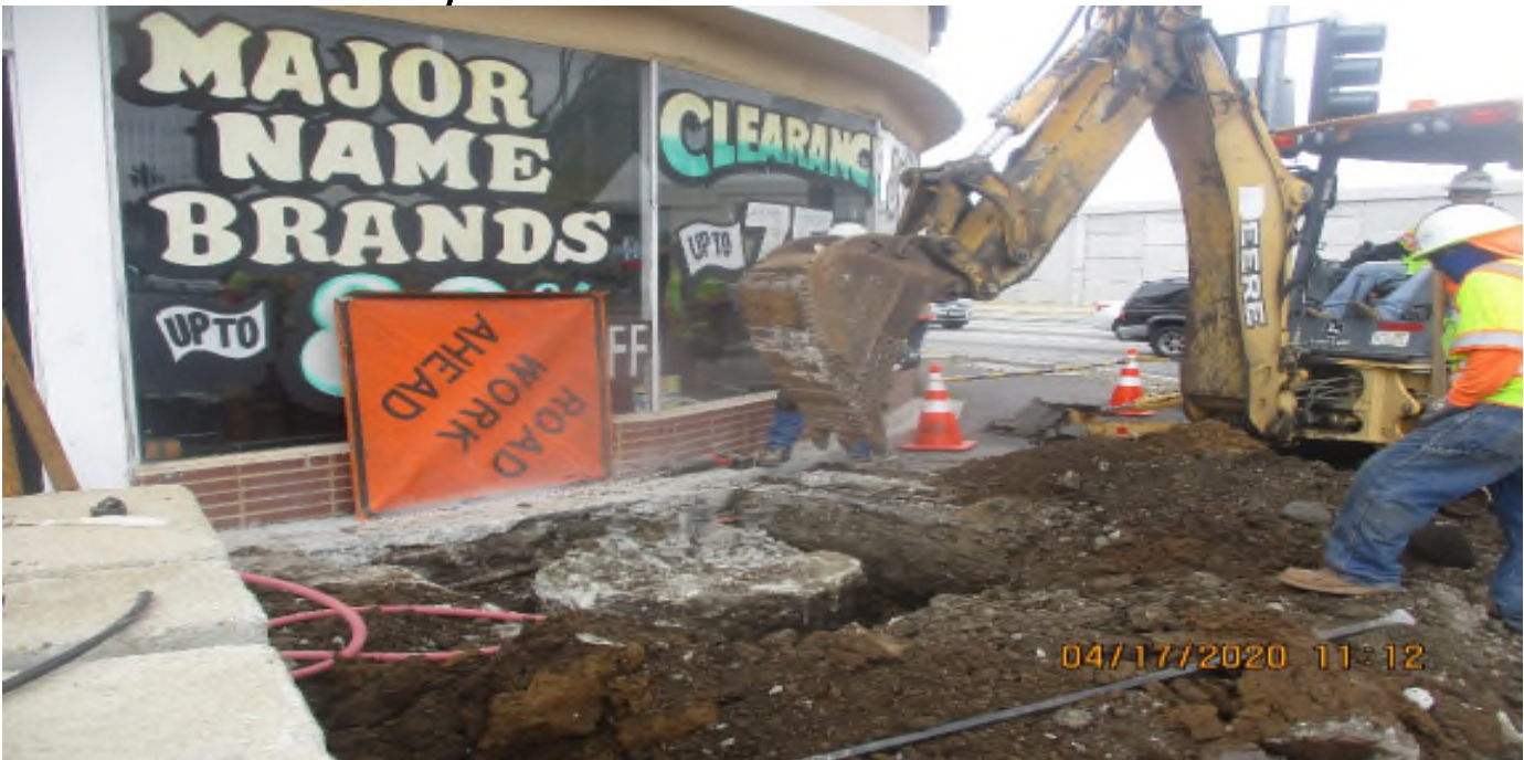
Florence/Brea – Select Electric Removed existing TS foundation at S/E corner of La Brea and Florence.
