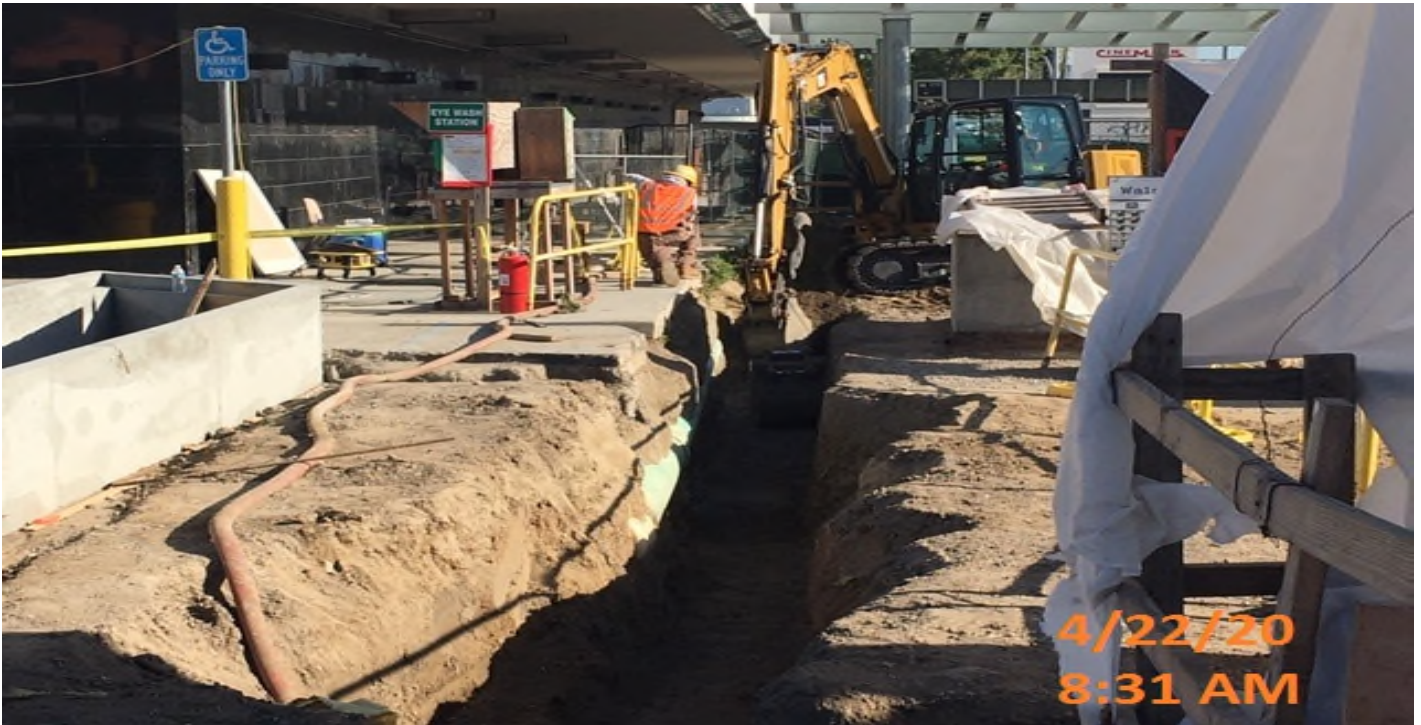
MLK STATION – Continue excavating for new 12” HDPE drainage pipe adjacent to Elevators 1&2 at the plaza level.
