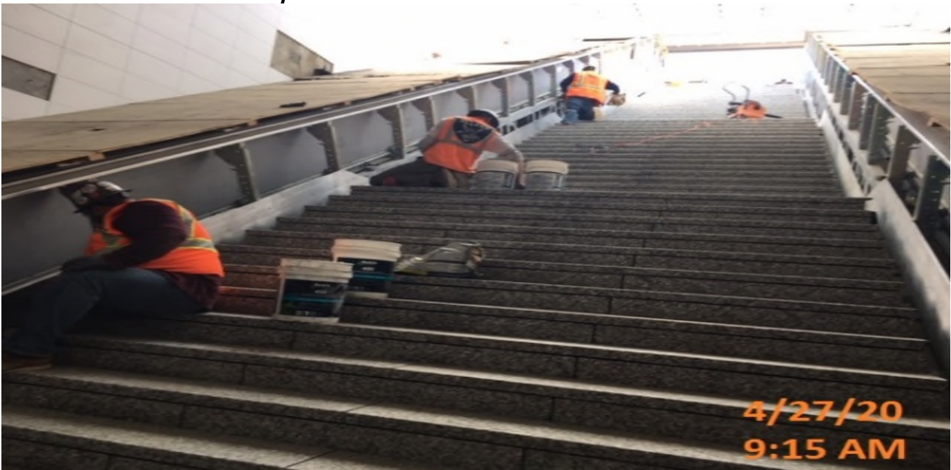
EXPO STATION – Continue granite runner section installation at the main entrance staircase of the plaza level.
