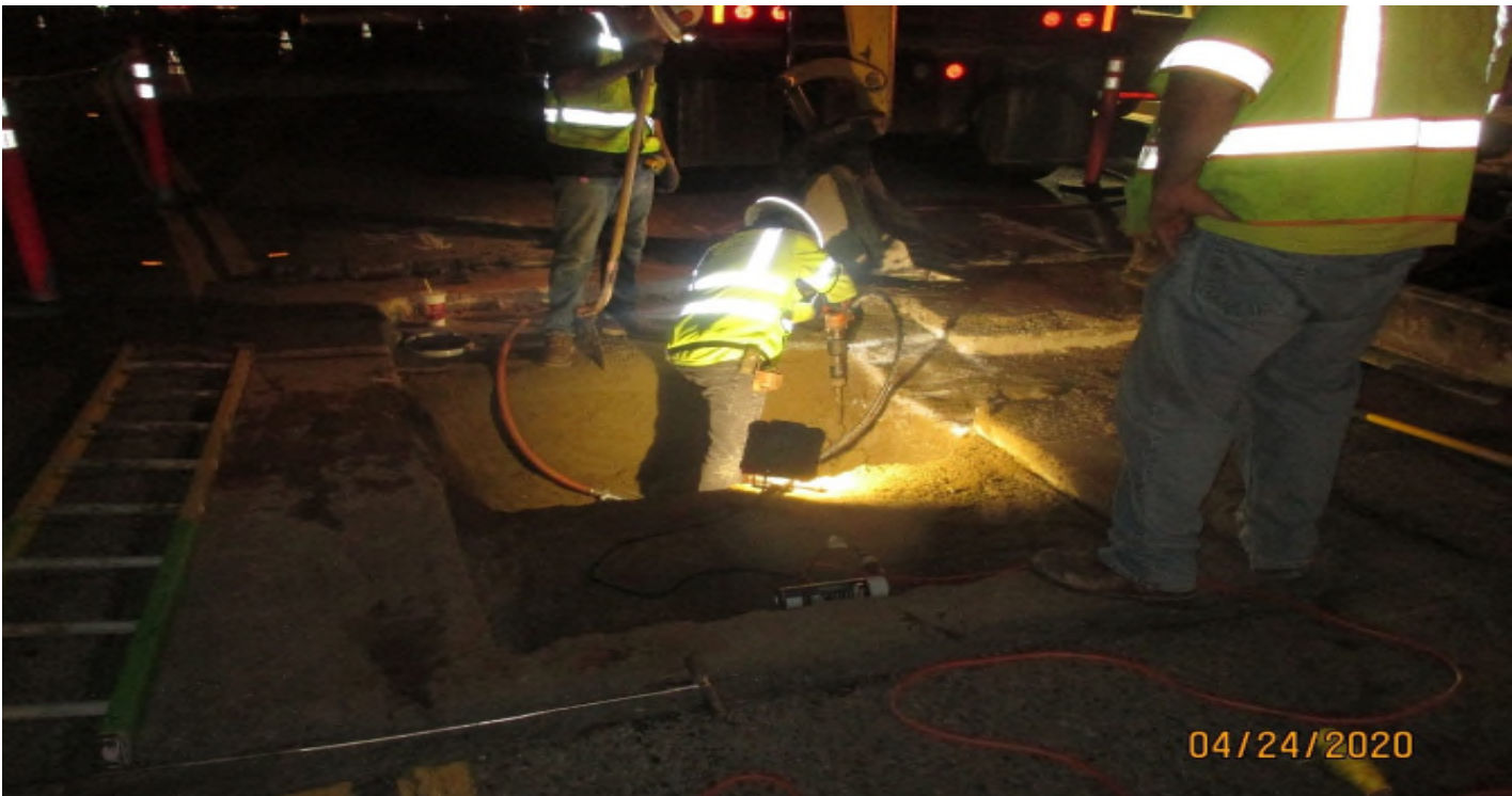
UG1- Excavating the fire line trench through slurry at the UG-1 south portal.
