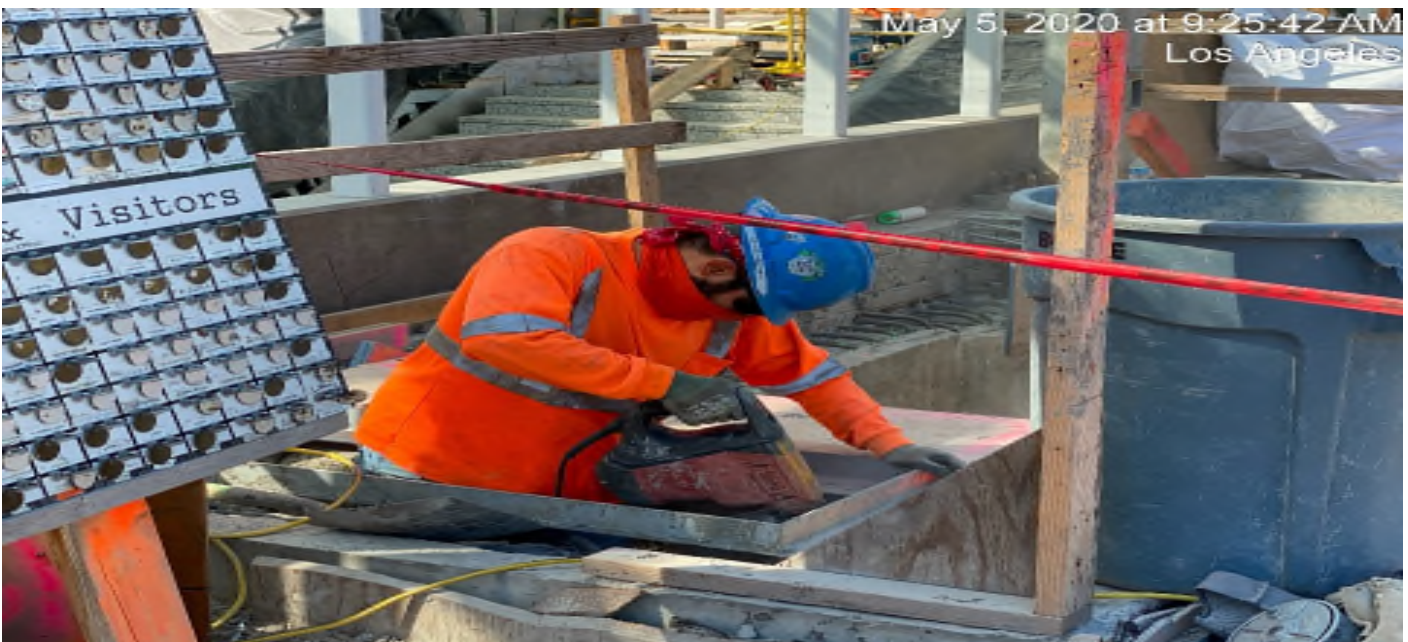
LEIMERT PARK STATION – Continue drilling and doweling for the north emergency exit hatch doors at the plaza level.
