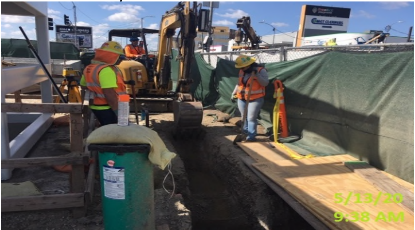
EXPO – WSCC crew trenching for Select Electric to lay 1' conduit for sidewalk lighting.
