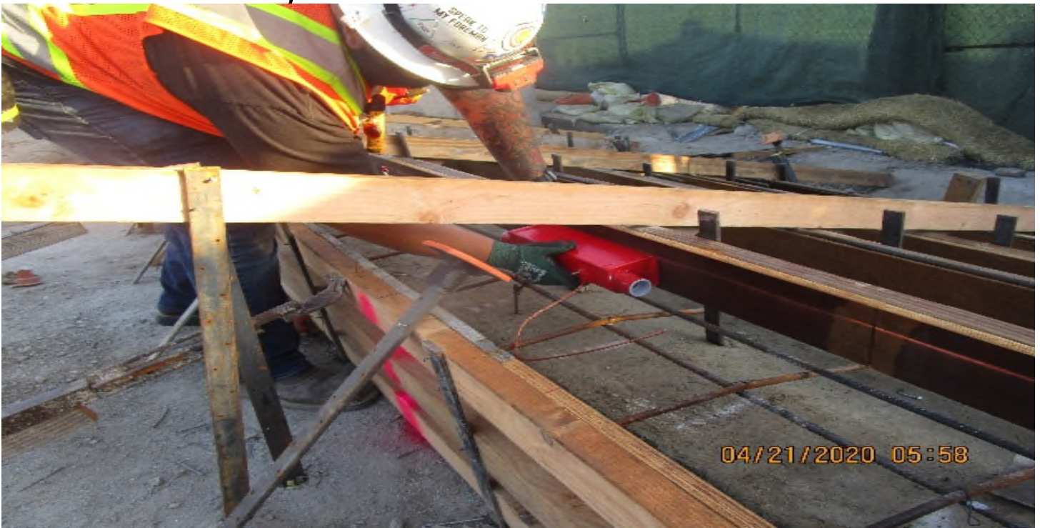
Crenshaw/Vernon - STA 363+00 TK#3 – new 22.7' rail plug delivered on site for T&M work Vernon Station
