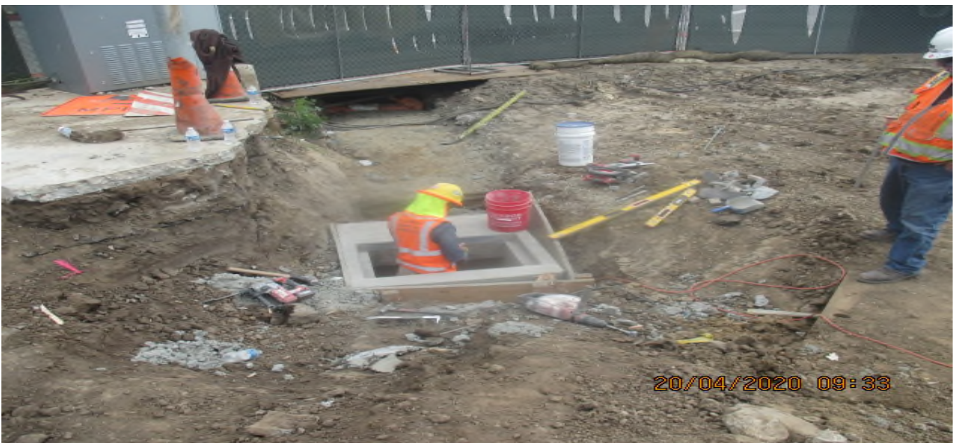
UG3 – Continue excavation for the new sidewalk/driveway installation on the southwest corner of 67th St and Crenshaw Blvd. 3/20/20
