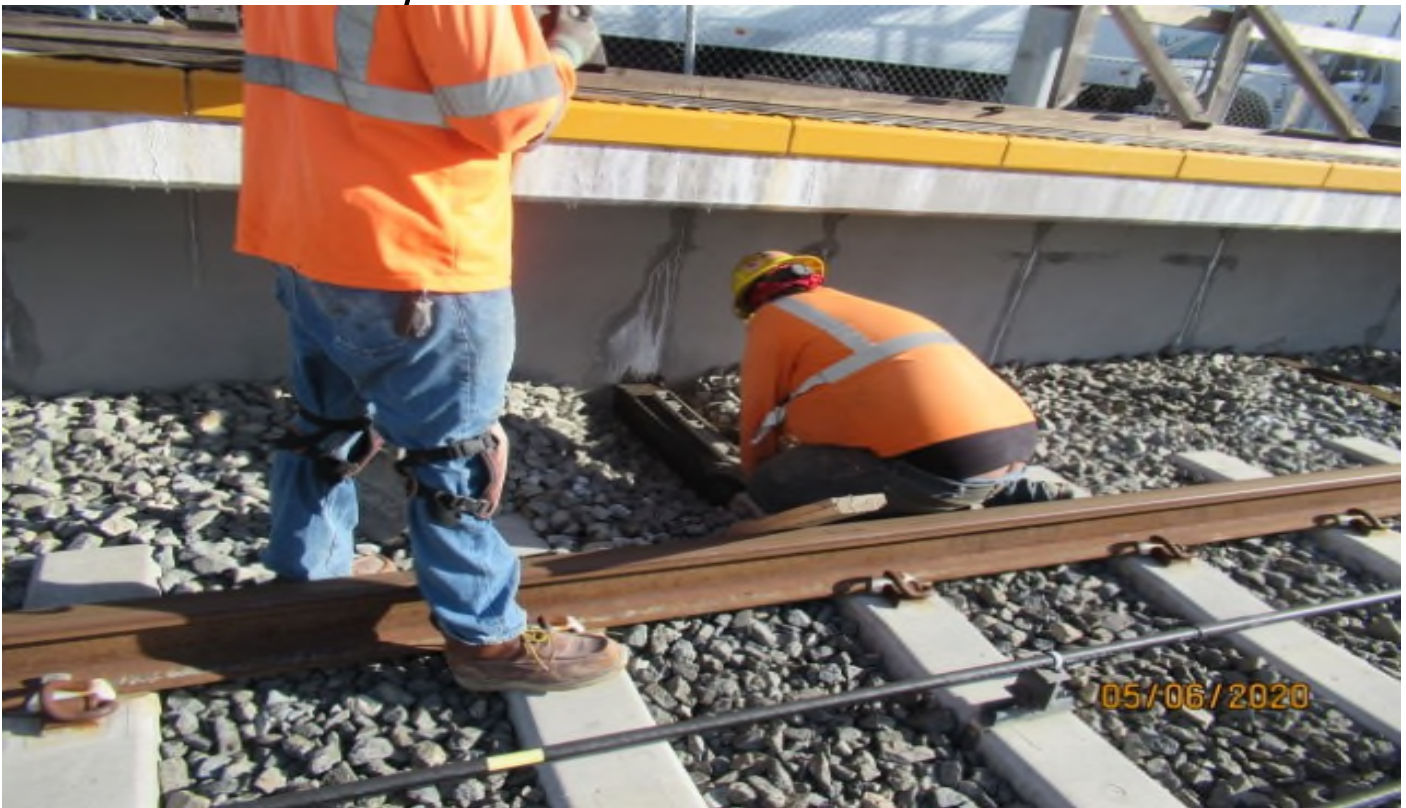
HINDRY STATION- WSCC leveling treaded timbers on SB #3 track, at Hindry station platform rework.
