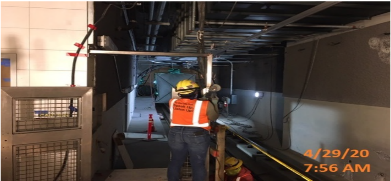
MLK STATION – Installing header and grinding welds for the south end platform end gates.
