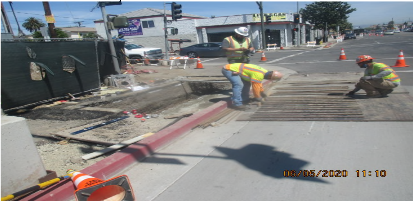
UG3 – Continue installing rebar mat for the street light foundation on the southwest corner of 67th St and Crenshaw Blvd. 5/6/20
