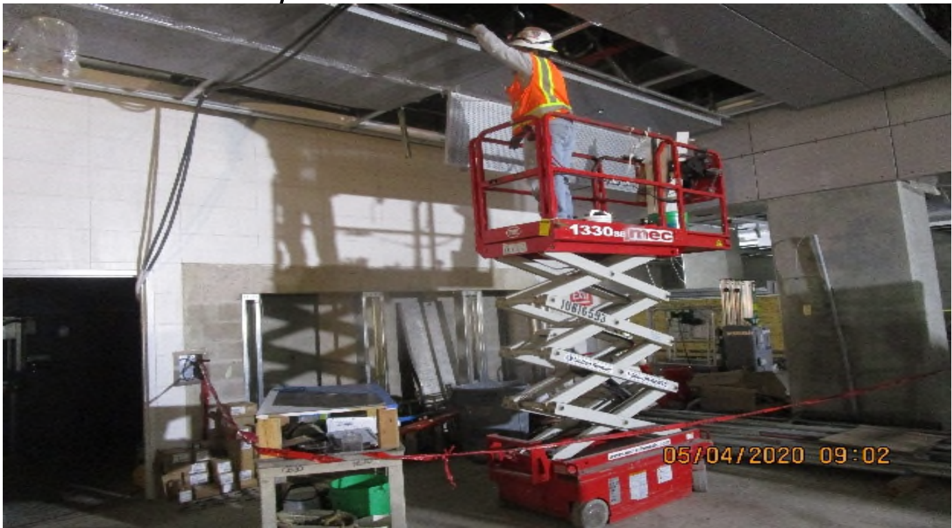
Crenshaw/Vernon - Vernon Concourse, Free Area C129, continued rough in of AL1A-Lumium brand lighting fixtures at light pockets
