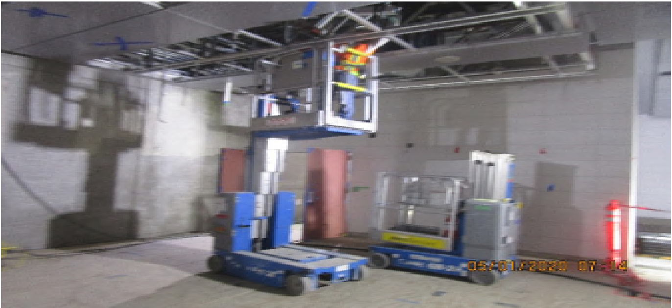
MLK STATION – Resume installation of ceiling light fixtures at the concourse level.
