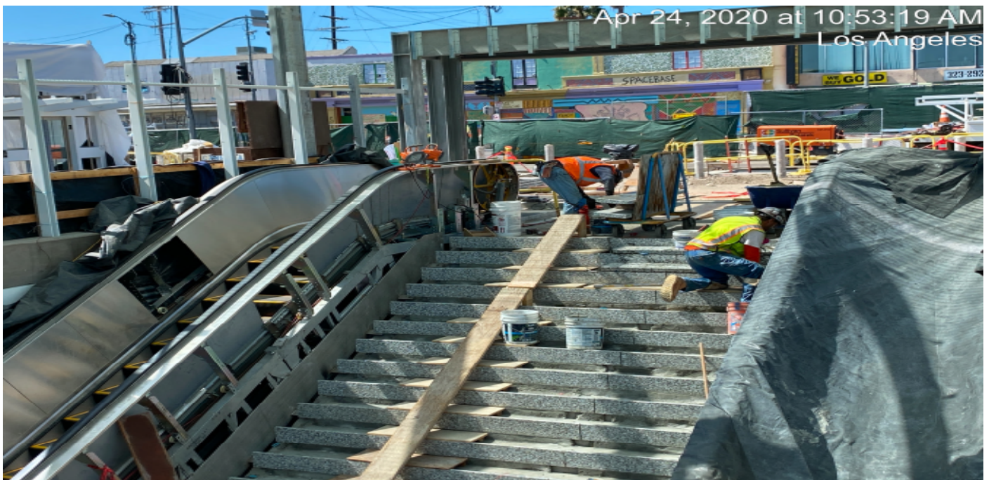
LEIMERT PARK STATION – Continue granite thread and riser installation at the main stair case landing of the plaza level.
