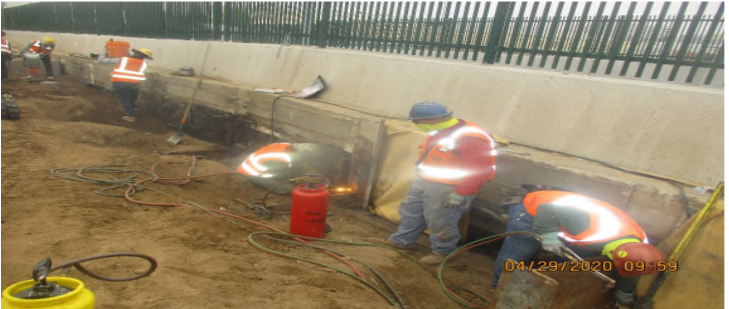
UG1 - WSCC Cut and remove 18" of soldier beams at 104th and UG-1
