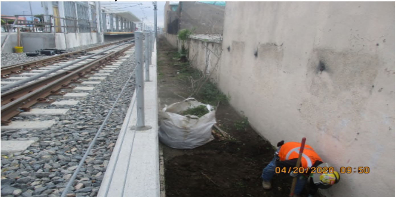
Florence/West – WSCC Clearing and grubbing in swale area at ballast wall at West Station.
