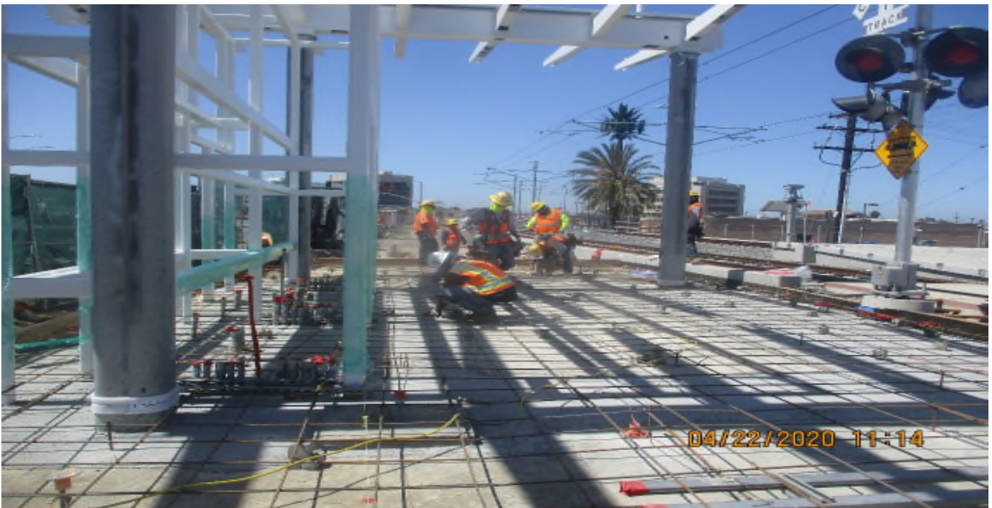
Florence/Brea – Complete forms for concrete at south ticket pavilion at La Brea Station.
