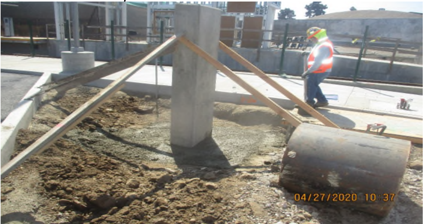
Florence/West – WSCC Placing concrete pace of generator pedestal at West Station parking lot.
