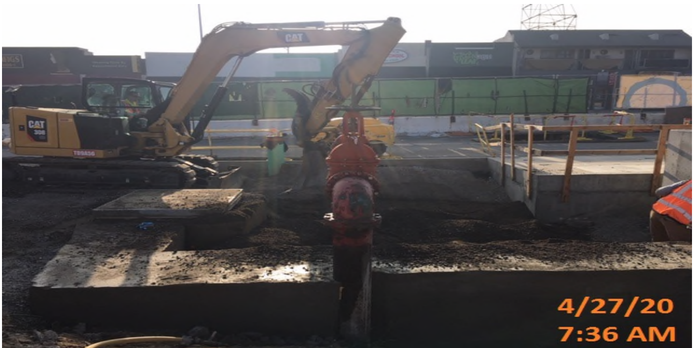
MLK STATION – Backfilling areas around the water backflow preventer valve on the east side of the plaza level.
