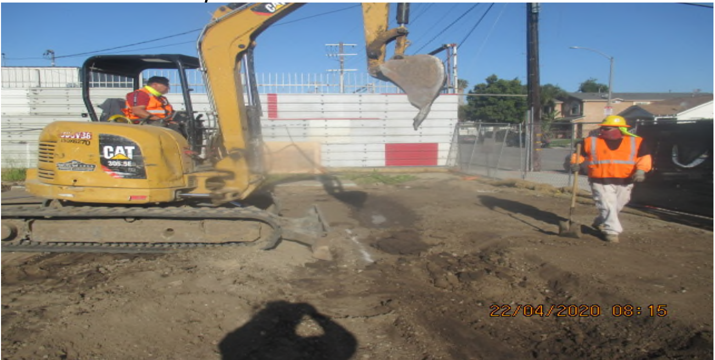
UG3 – Continue excavating for the culvert swales for the drainage structure on the north east corner of Victoria Yard. 4/22/20
