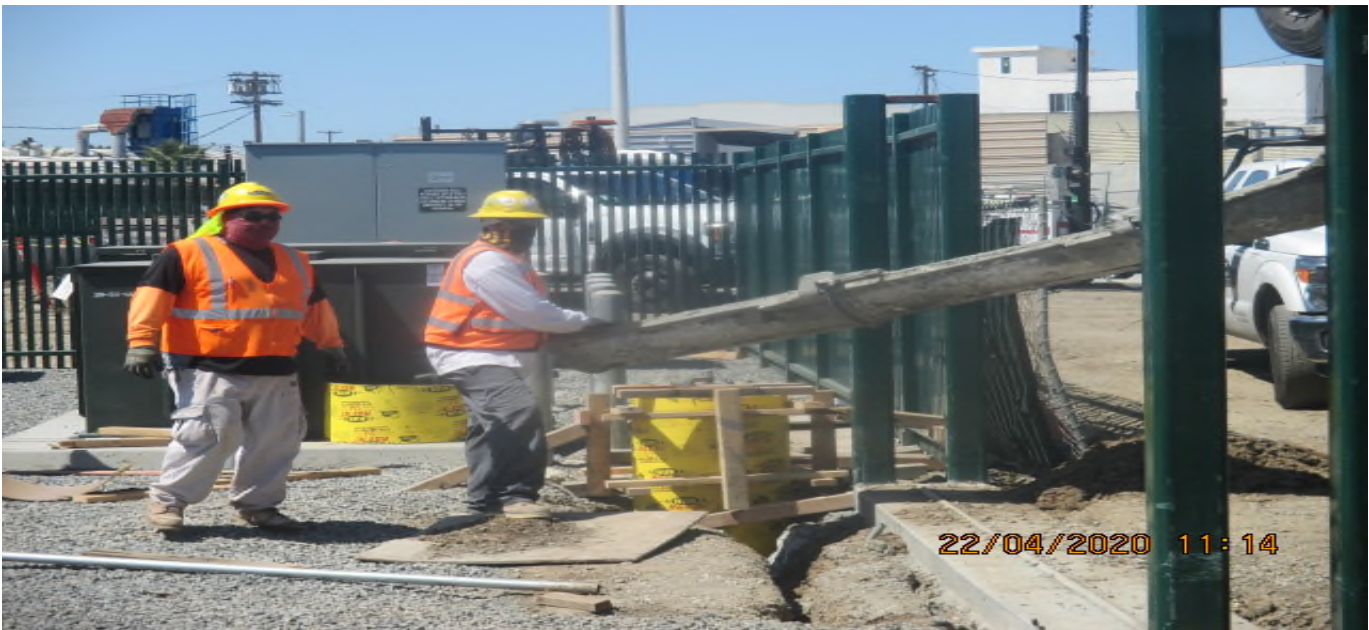
UG3 – Placing concrete on the light pole foundations on both sides of the Auxiliary Power Bungalow at Victoria Yard.
