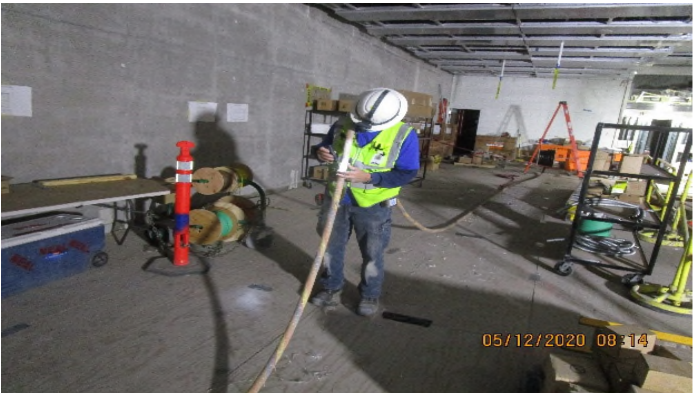
Crenshaw/Vernon - Vernon concourse, Elevator #4, Re-pulling main traveler wiring harness do to 1st traveler to short in length-Rework
