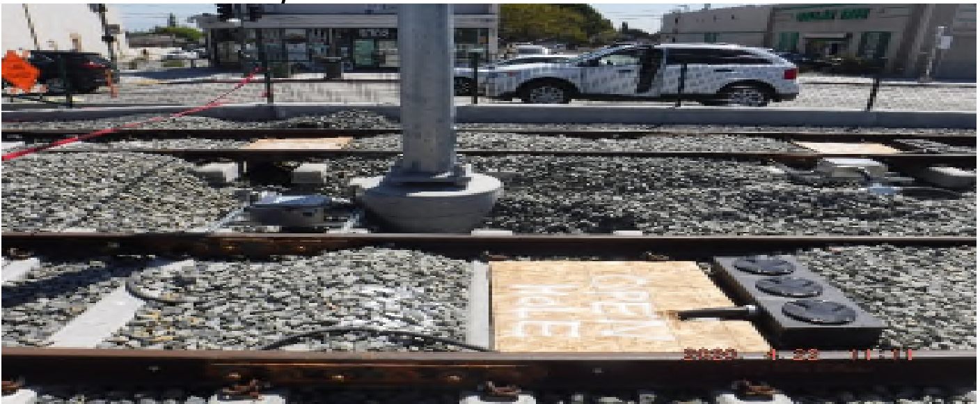
57 th Street - STA 329+75 TK#3/SB looking east – system work with track structure disturbance south of 57th St around/next to OCS #1258 as of 4.22.2020 – PUNCH LIST
