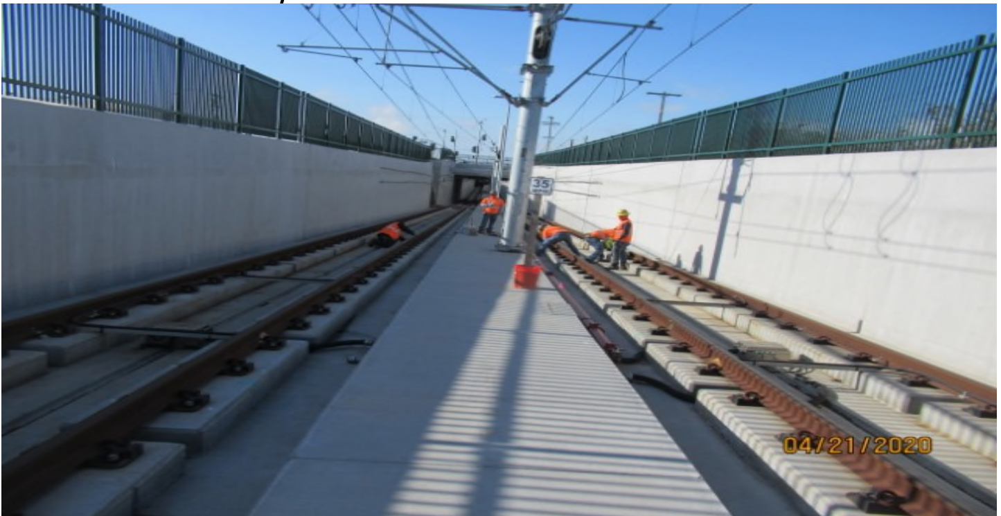
UG - 1 – WSCC crew in UG1 both NB & SB tracks, for install of epoxy on expansion joints (looking south) out of sequence
