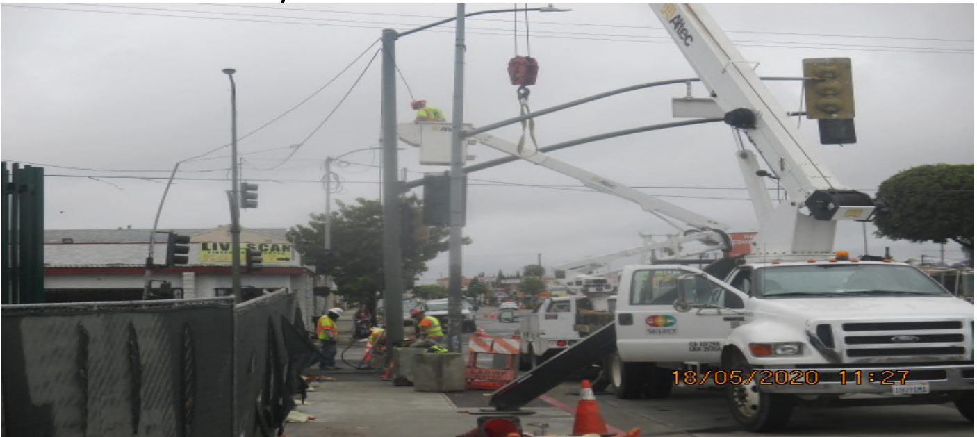
UG3 – Continue pulling power to pull boxes to supply runs for the street light pole on the southwest corner of 67th St and Crenshaw Blvd. 5/18/20
