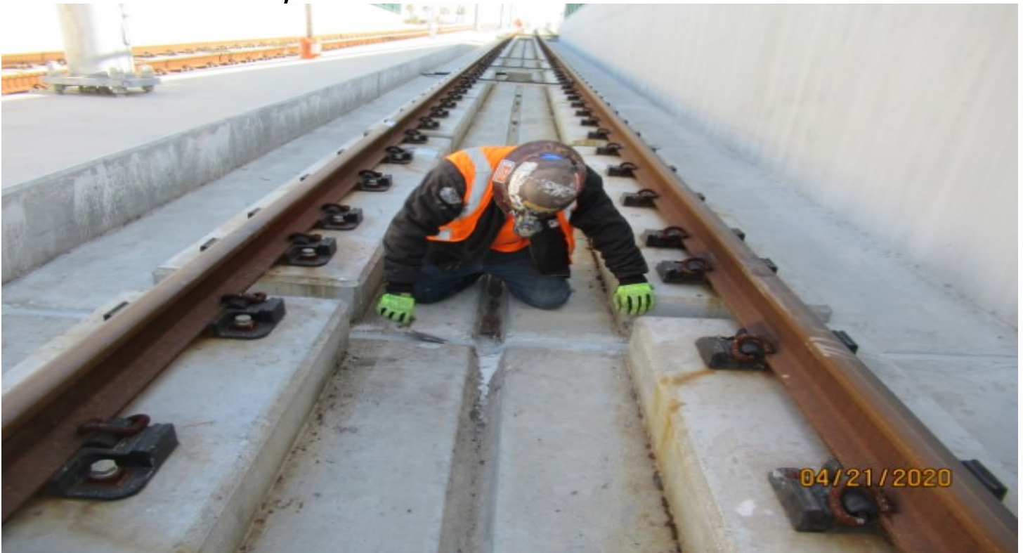
UG1 – WSCC placing epoxy on expansion joints in UG1 NB #4 track out of sequence work
