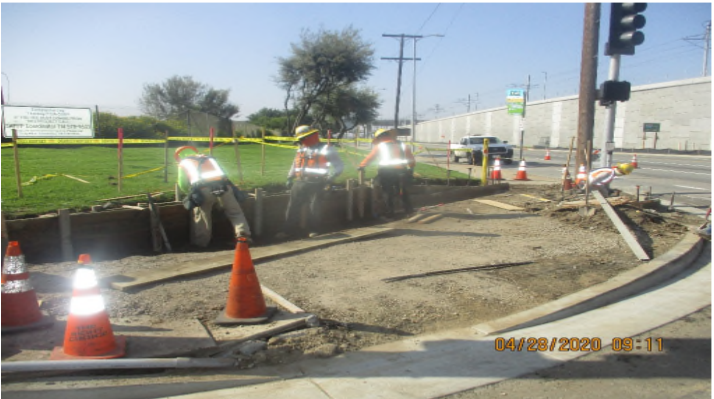
AVIATION/CENTURY- WSCC Form and place conc for small retaining wall at S,WCOR of 111th and Aviation
