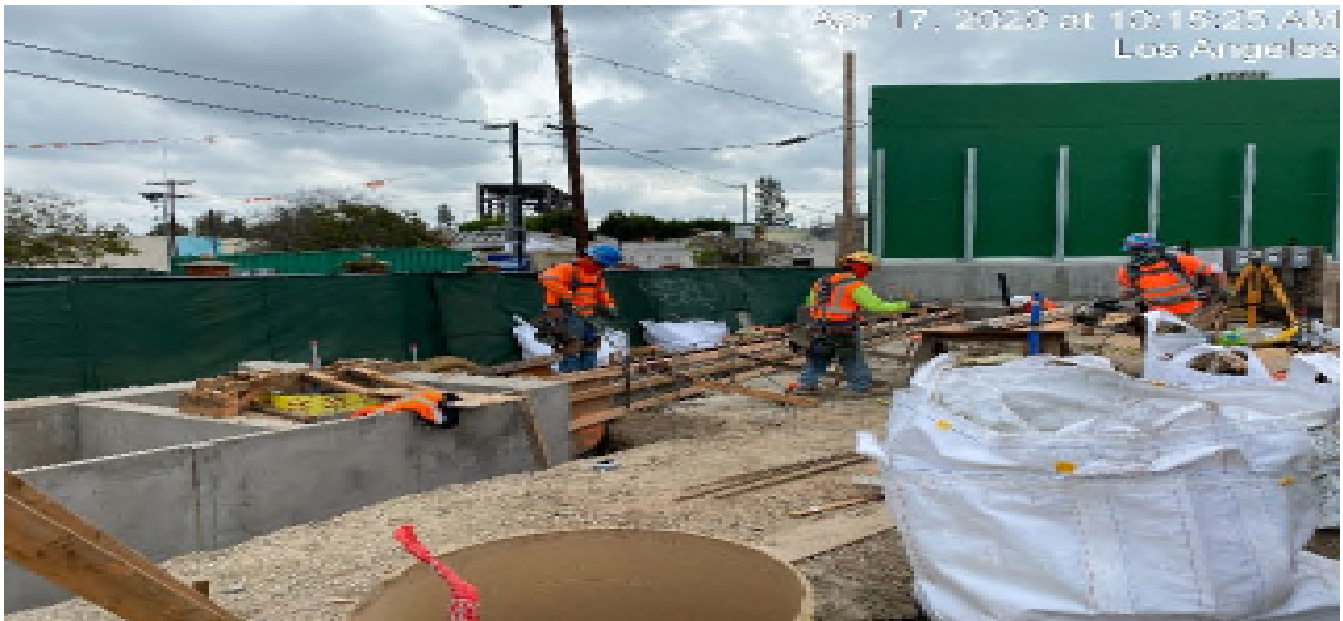
LEIMERT PARK STATION – Continue tunnel fan damper section installation for the sound attenuator for EVF-6-102 in the North Fan Room C – 142 of the concourse level.
