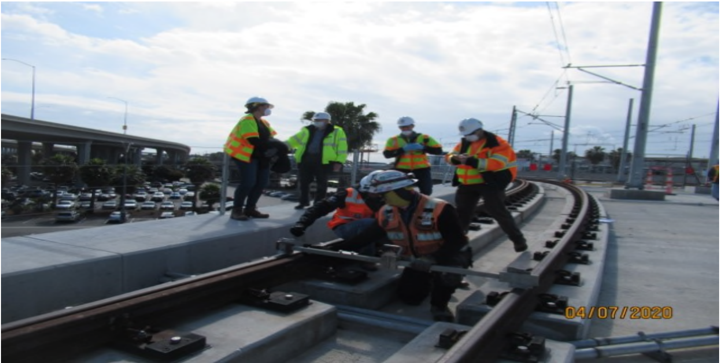
Green Line underpass – Metro & HCC cross referencing rail templates that matched for rail profile radius for HRC-CPF on NB1300 track GL Wye STA 12+56 (looking southeast)
