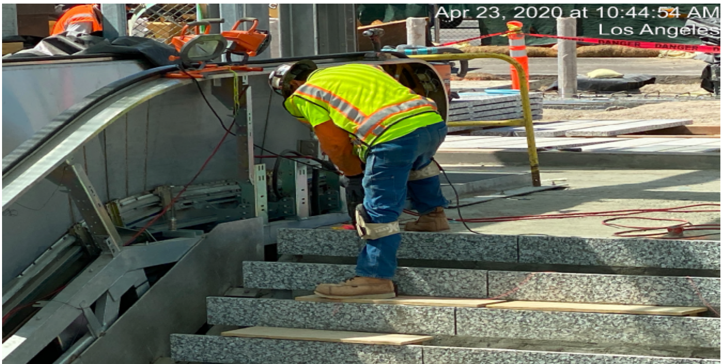
LEIMERT PARK STATION – Continue granite thread and riser installation at the main stair case landing of the plaza level.
