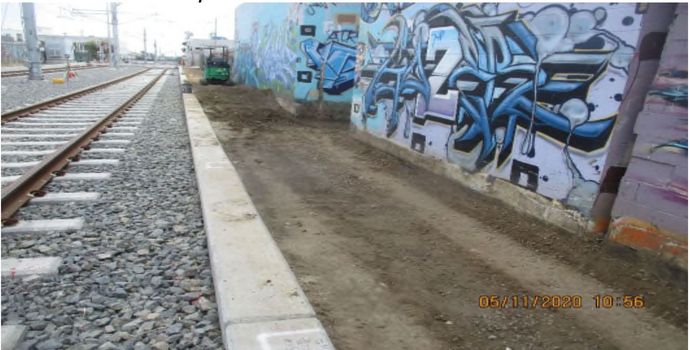
Florence/West – WSCC Make grade for swales on both ROWs east of West St.
