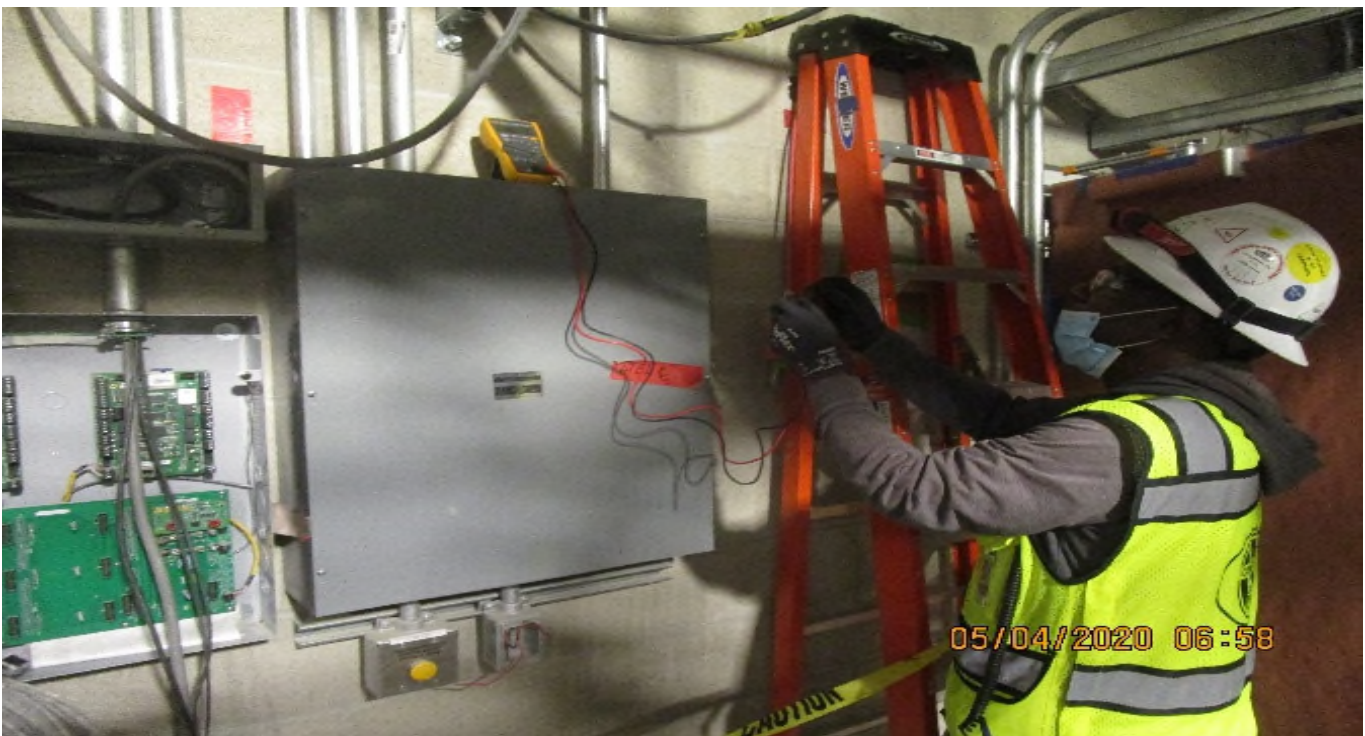
MLK Concourse, TC&C Room C113, Continued continuity testing of 1 pair #14 fire alarm strobe wiring.
