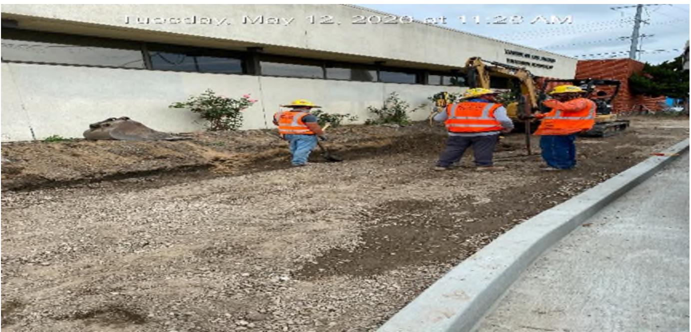
EXPO STATION – Excavating trench for new sidewalk/curb installation on southbound Crenshaw Blvd between Exposition Blvd and Rodeo Blvd.
