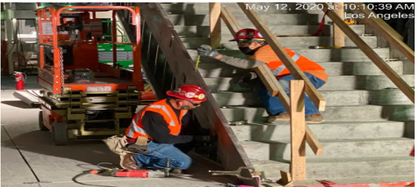
LEIMERT PARK STATION – Installing metal steel framing at the underside of stairwells 3&4 at the platform level.
