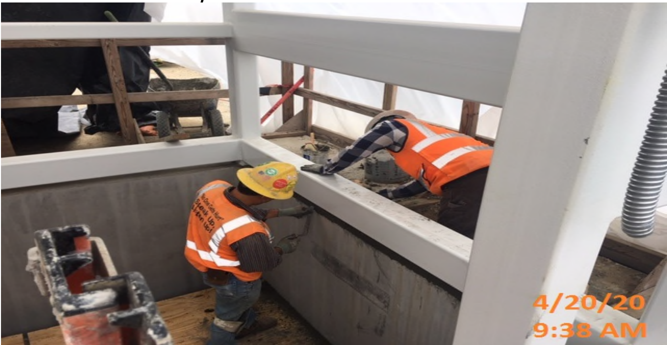
EXPO STATION – Patching and surfacing walls for Elevator shafts 1&2 at the plaza level.
