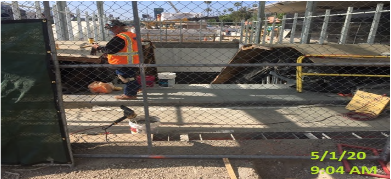
MLK STATION – Grouting pavers at the top landing of the main entrance structure of the plaza level.
