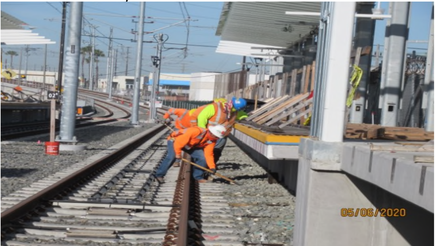
HINDRY STATION- WSCC hand dressing shoulder ballast & leveling treaded timbers on #3SB track throughout Hindry station platform (looking south) rework
