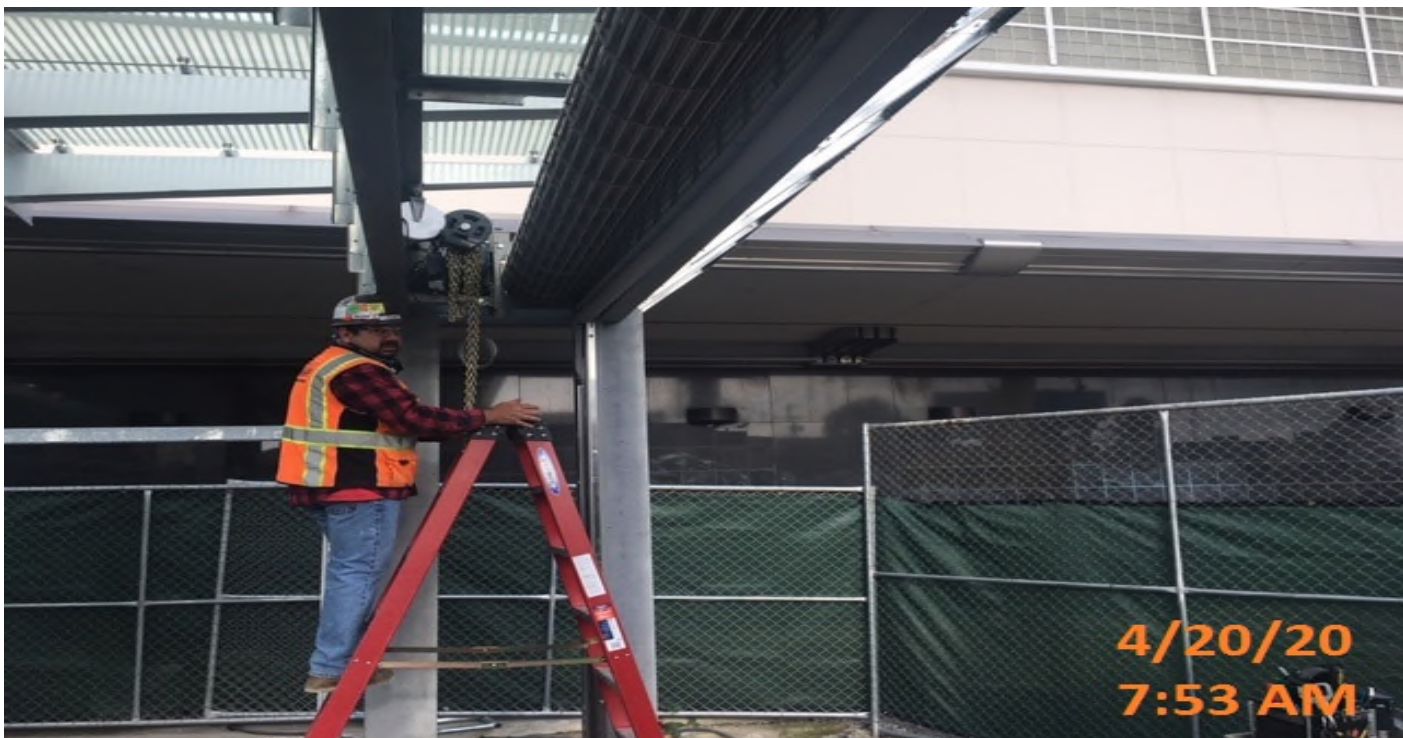
MLK Station - Installing motor for the overhead coiling grille door to the main entrance canopy at the plaza level.
