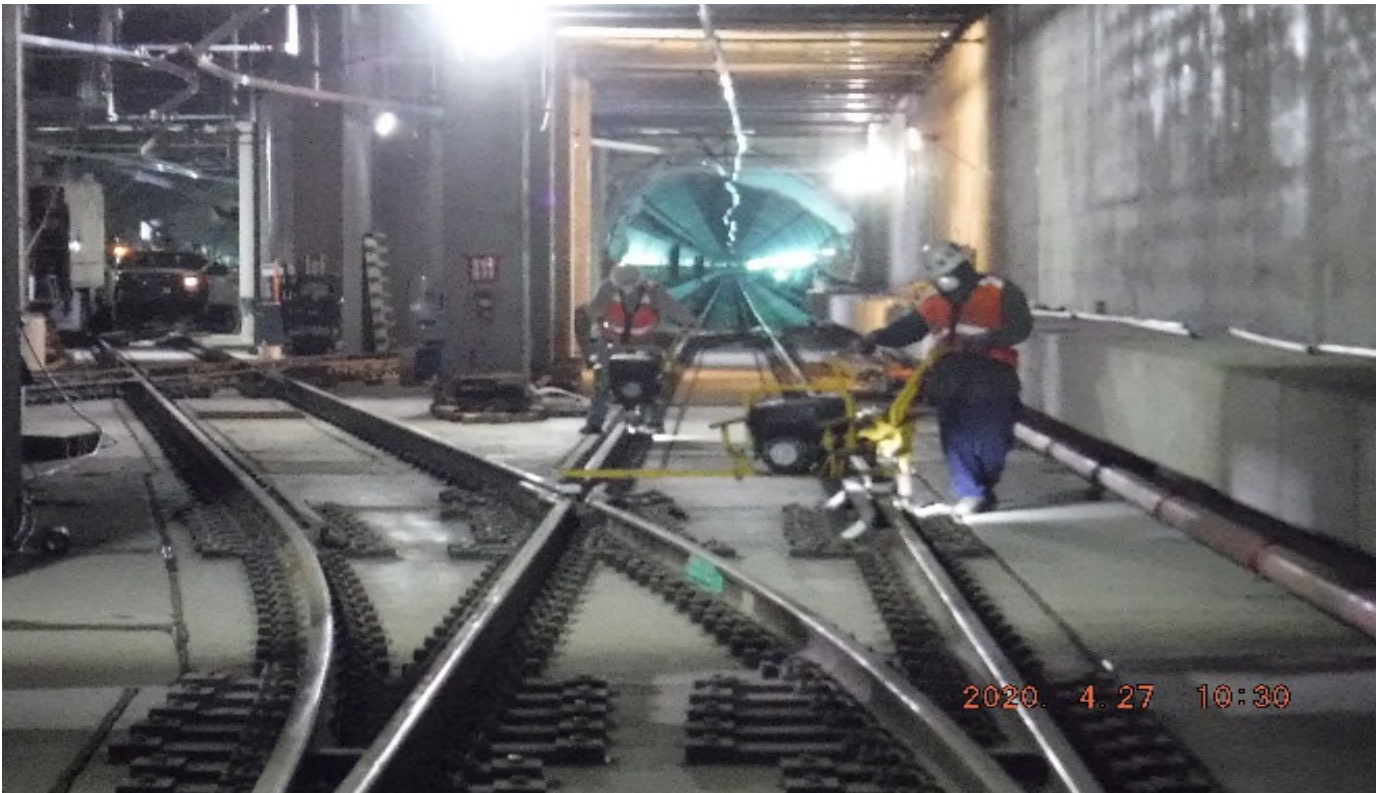
UG-4- STA 444+39 TK#3/SB looking south – torque DF fasteners between 8X1RH XO & 8W1LHXO – UG4 Exposition Station
