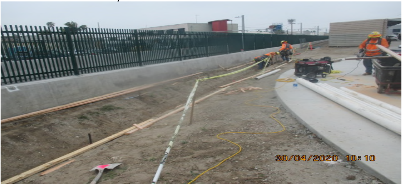
UG3 – Building forms for the culvert drainage system installation along the southbound barrier wall at Victoria Yard. 4/30/20
