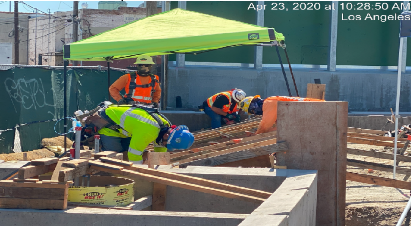
LEIMERT PARK STATION – Continue formwork for the planter stair risers on the northwest section of the plaza level.
