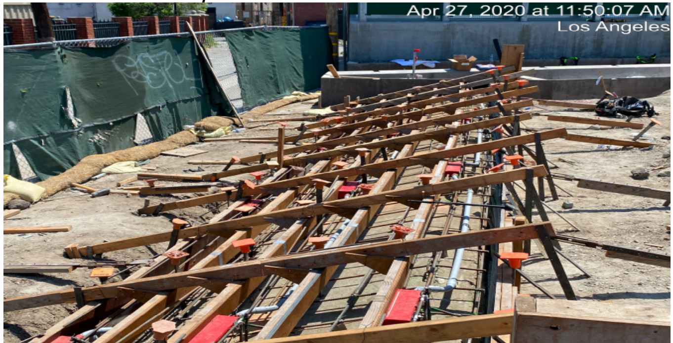
LEIMERT PARK STATION – Continue formwork for the planter stair risers on the northwest section of the plaza level.
