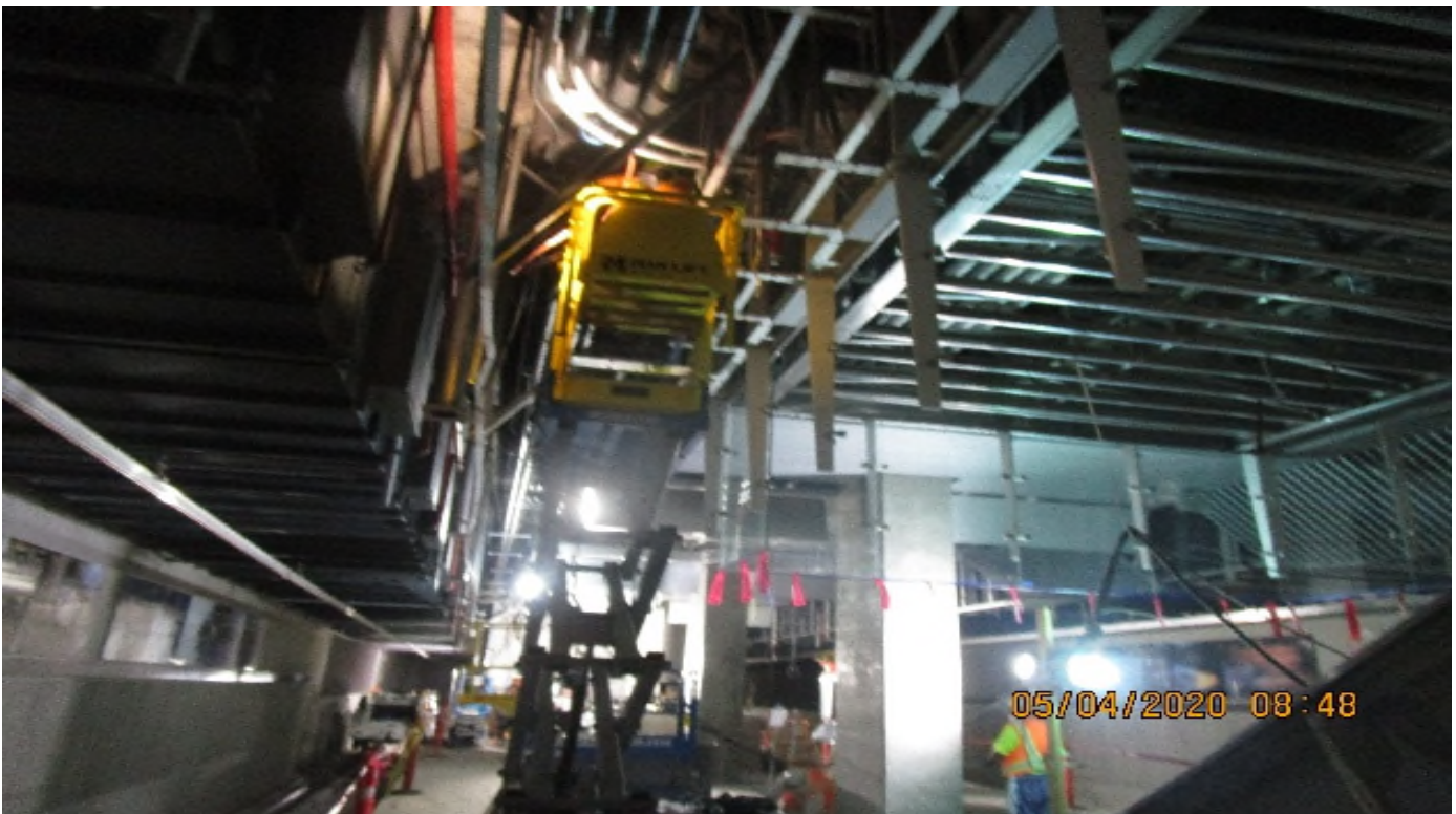
Crenshaw/Vernon - Vernon Platform, NB, begin overhead bonding Radiax GRC (5) 2" GRC with #2 7-strand bare copper grounds
