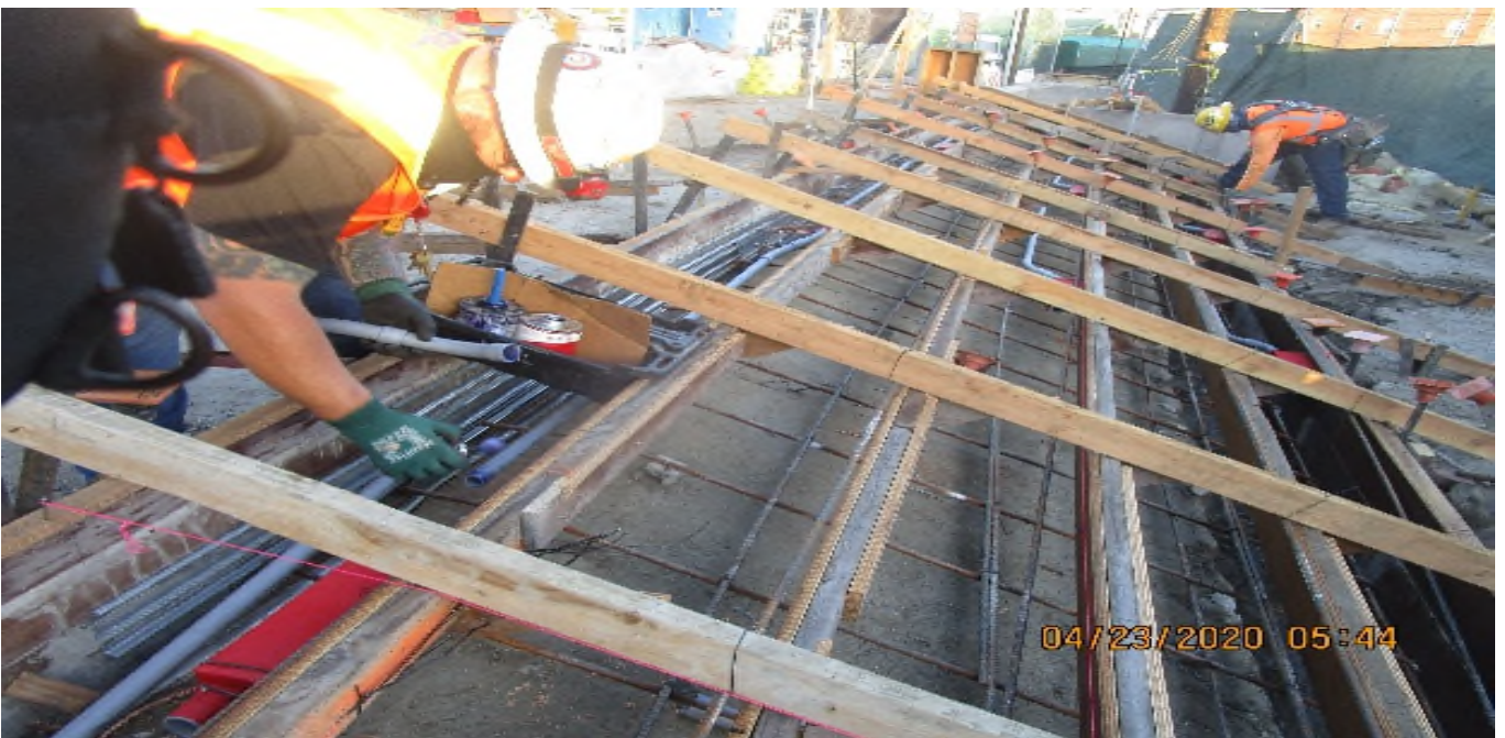
LEIMERT PARK STATION – Continue embedded and ramp lighting fixture installation for the planter stair risers on the northwest section of the plaza level.
