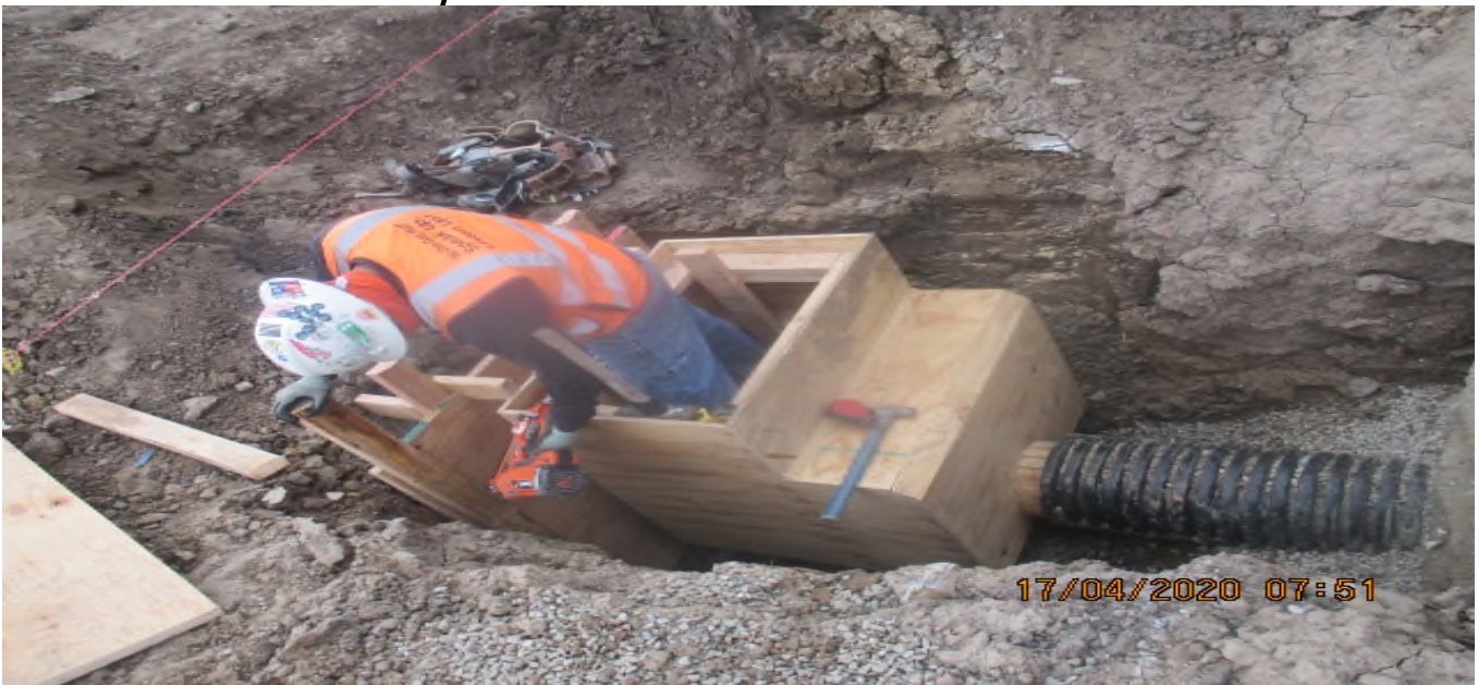
UG3 – Building forms for the drainage structure connecting to Catch Basin #1 on the north east corner of Victoria Yard. 4/17/20
