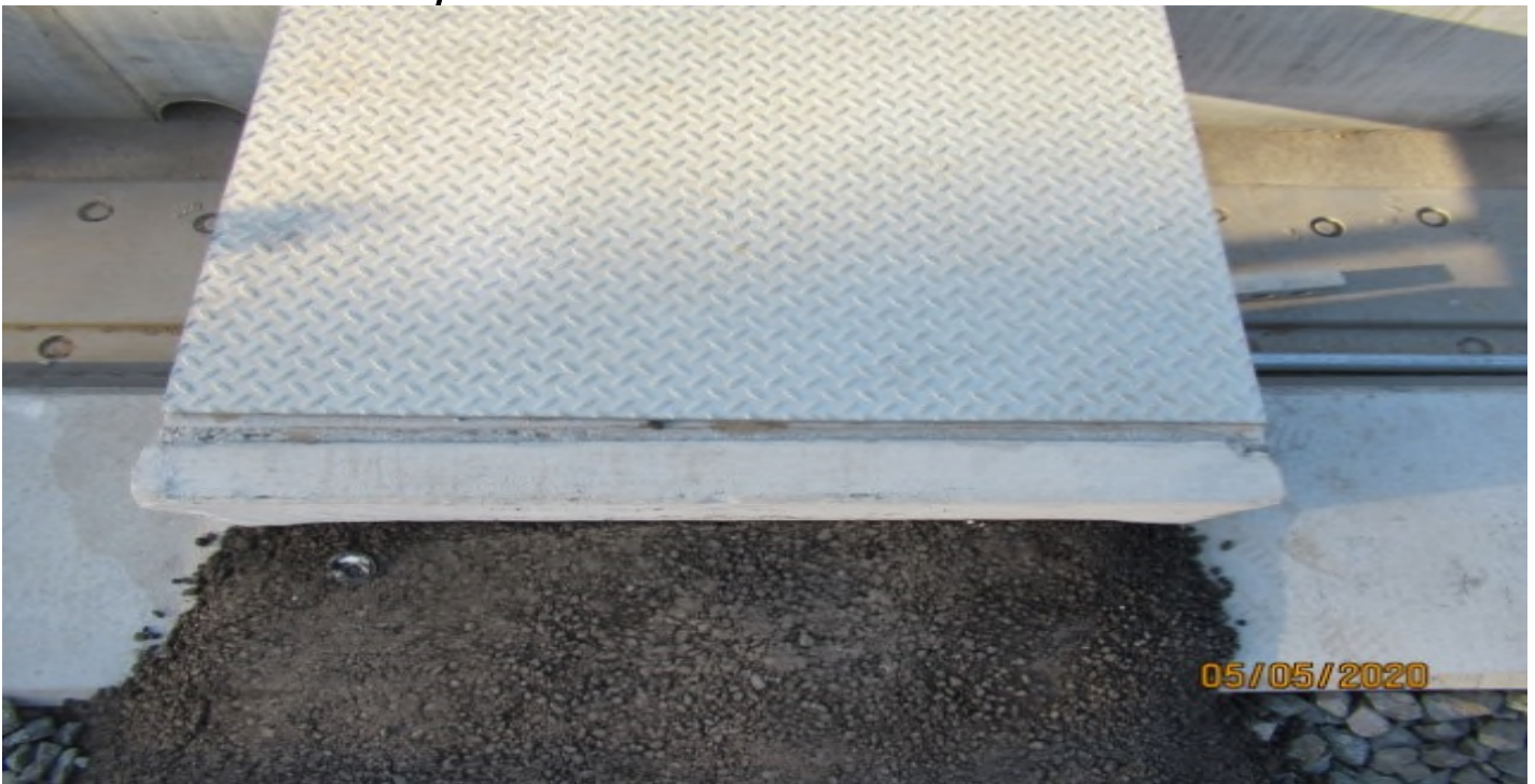
AVIATION/CENTURY - Emergency Walkway crossing at edge of DF track on Century/Aviation bridge STA 74+72.
