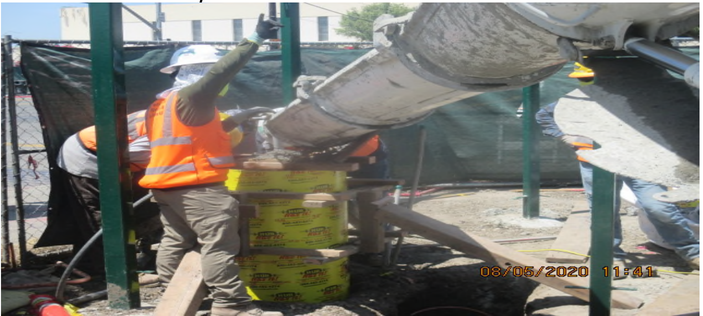
PARK MESA – Placing concrete for the light pole foundations at the northeast corner of TPSS#7 on 60th St & Crenshaw Blvd. 5/8/20
