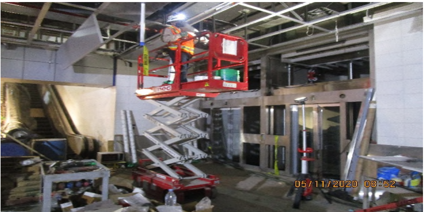
LEIMERT PARK STATION – Continue installing ceiling light fixtures at the concourse level.
