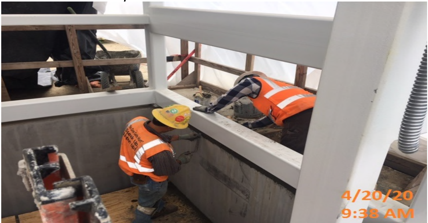
Crenshaw/Expo - EXPO – WSCC finishers patching and surfacing walls of elevator shaft #1 and #2.
