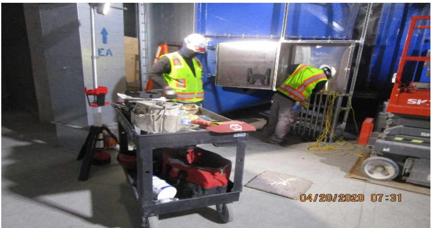
Crenshaw/MLK - MLK, Emergency Fan room (S) C102, EVF-7-121, continued rough in 36"x36"x12" PB & begin FRP to control panel
