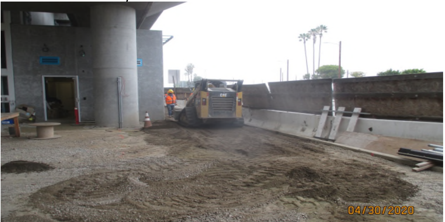
AVIATION/CENTURY- Placing base on the east side of the Aviation Station service building.
