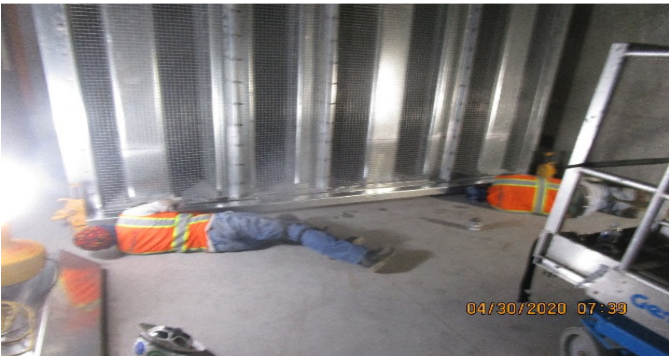
MLK STATION – Began bird screen protection and hardware support installation to TFD-7-322 in the North Tunnel Vent Plenum C – 140 of the concourse level.
