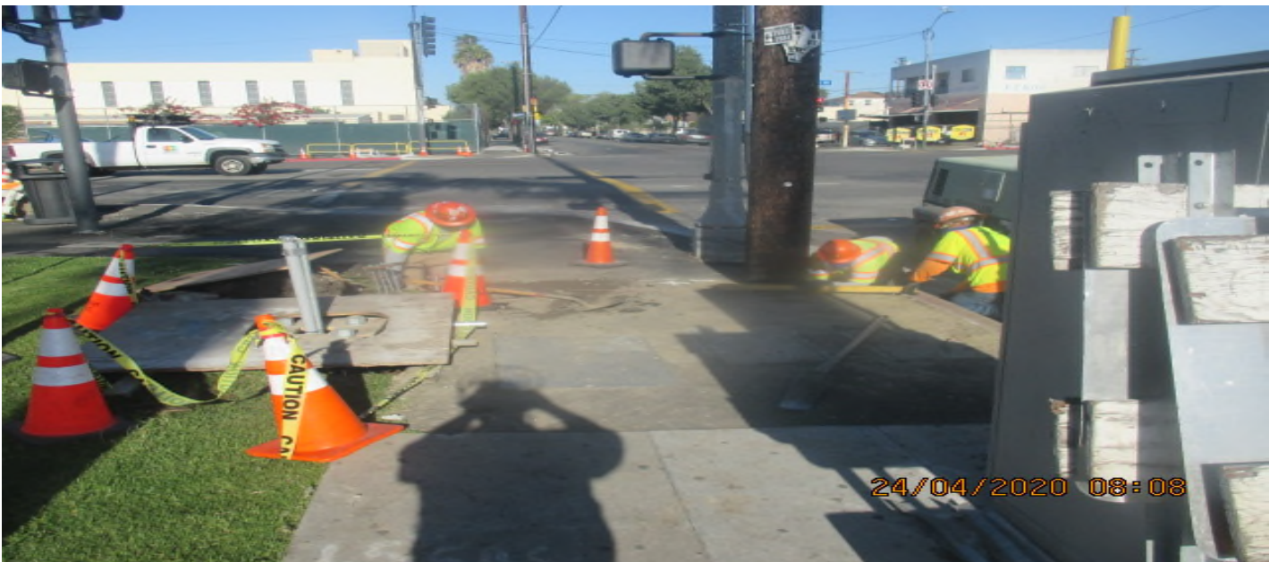
PARK MESA – Anchoring the generator to the housekeeping pad at TPSS#7 on 60th St & Crenshaw Blvd.
