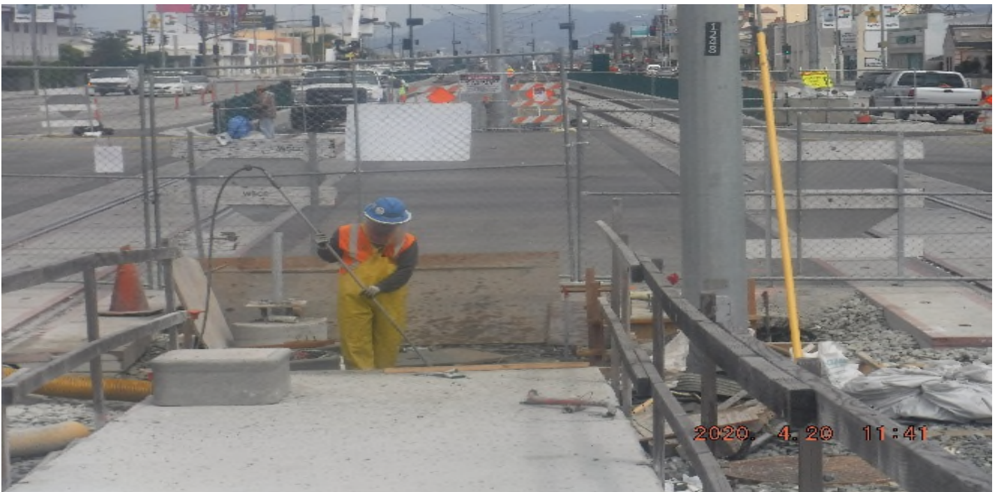
Crenshaw / Slauson - STA 323+00 TK#4/NB looking north – vacuum pole foundation excavation north end Slauson Station – PUNCH LIST
