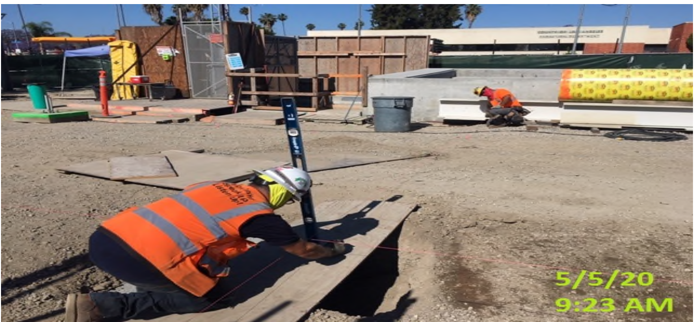
EXPO STATION – Adjusting and laying out for plaza lighting measurements at the plaza level.
