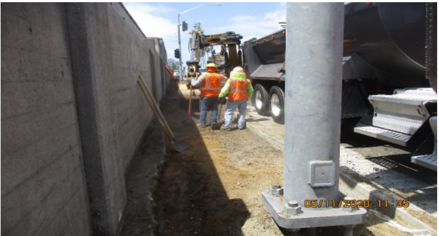
Florence/High St. - WSCC Cut and make grade for SWK pour at EB Florence and High St.
