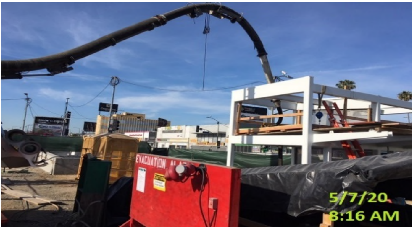
EXPO – Badger pumping water out from elevator jack shaft below pit at platform elevator #1 and #2.
