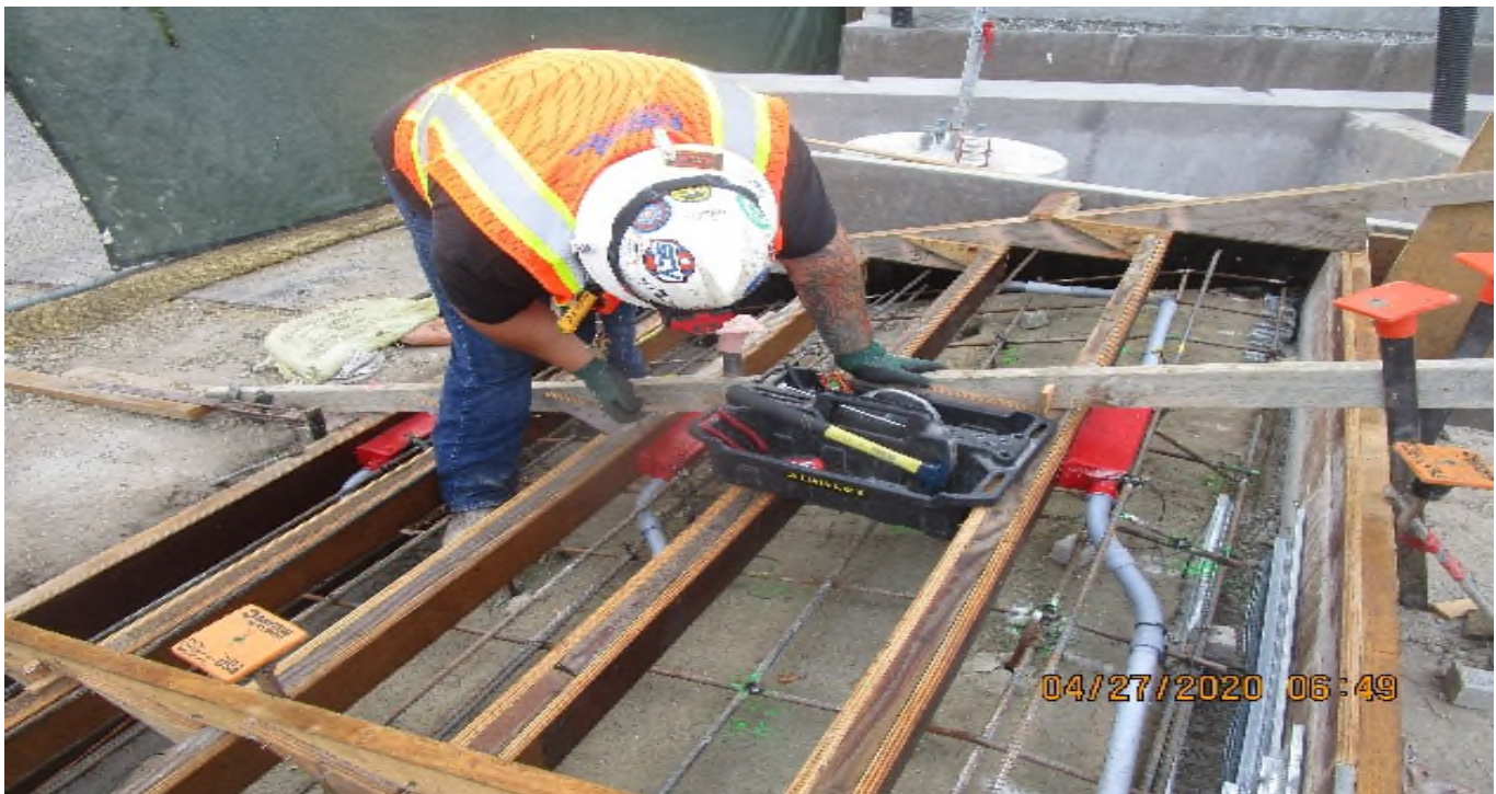
LEIMERT PARK STATION – Continue embedded and ramp lighting fixture installation for the planter stair risers on the northwest section of the plaza level.
