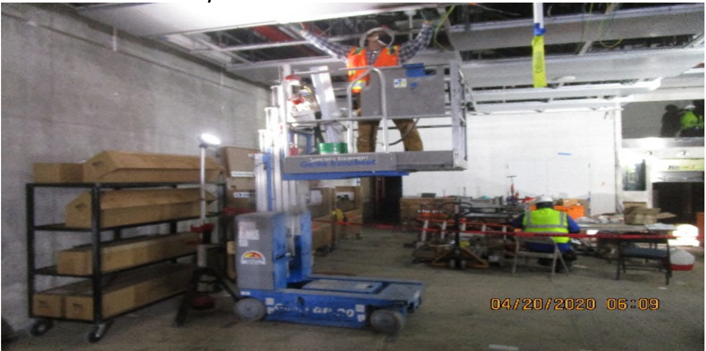
LEIMERT PARK STATION – Continue installing ceiling light fixtures at the concourse level.
