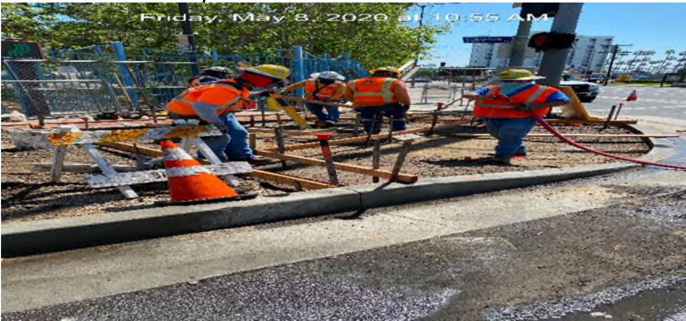
LEIMERT PARK STATION – Placing forms and concrete for new ADA ramp installation on the northeast corner of Vernon Ave and Crenshaw Blvd.
