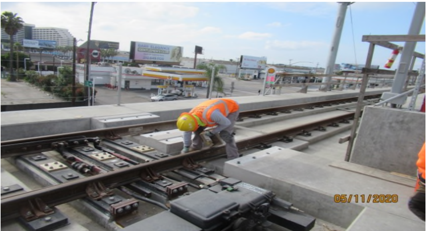
AVIATION/CENTURY - WSCC on NB #4 track STA 70+11 Century/Aviation bridge, repairing concrete foundations on emergency walkway's (looking southeast)
