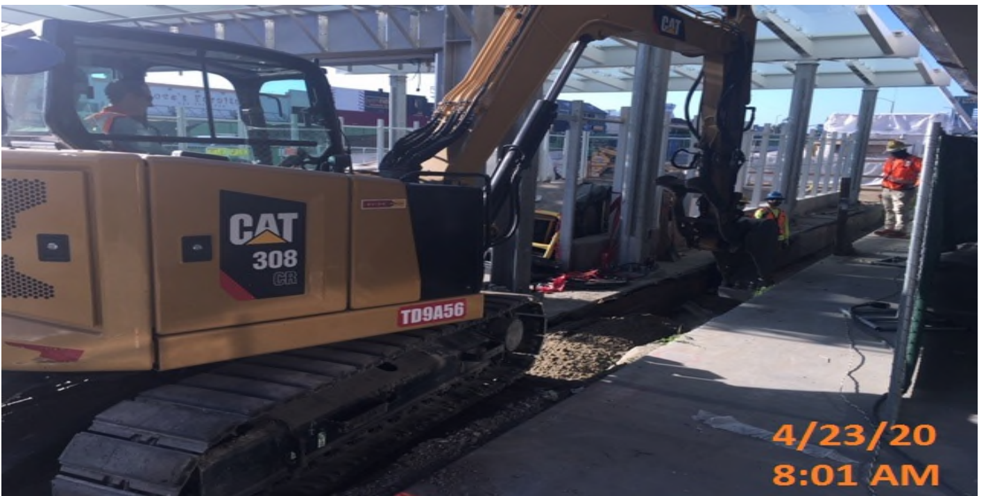
MLK STATION – Continue excavating for new 12” HDPE drainage pipe adjacent to the main entrance canopy structure at the plaza level.
