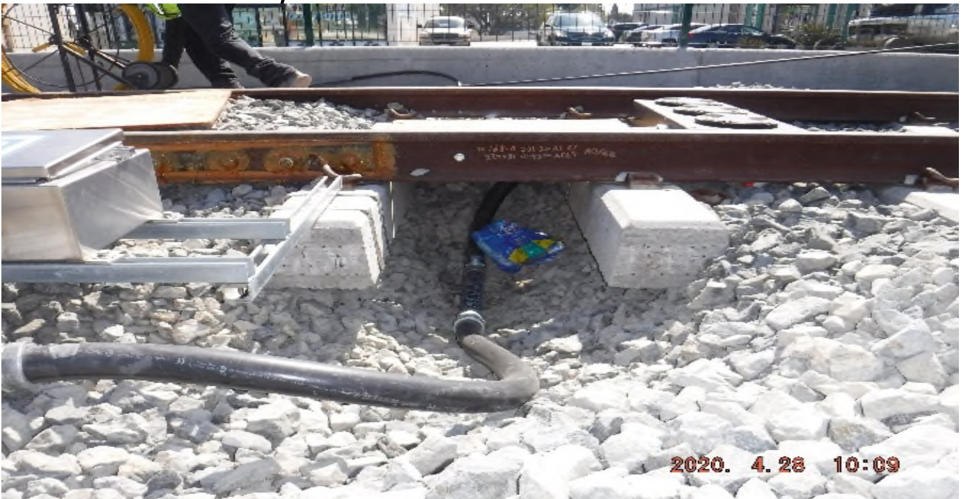
57 th Street - STA 329+75 TK#4/NB looking east – checking depth of system conduit imbedded in track structure south of 57th St.
