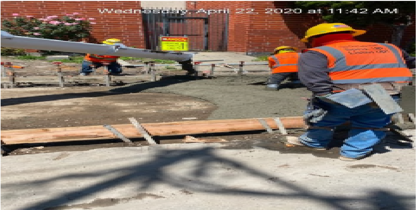
EXPO STATION – Placing concrete for new curb/gutter and bus pad installation on southbound Crenshaw Blvd between Exposition Blvd and Rodeo Blvd.
