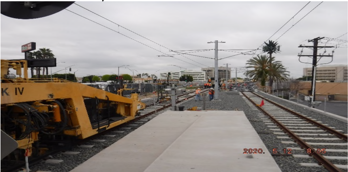
Florence/Brea - STA 208+00 TK#4/NB looking north – track geometry measurement south of La Brea Station before re-tamping
