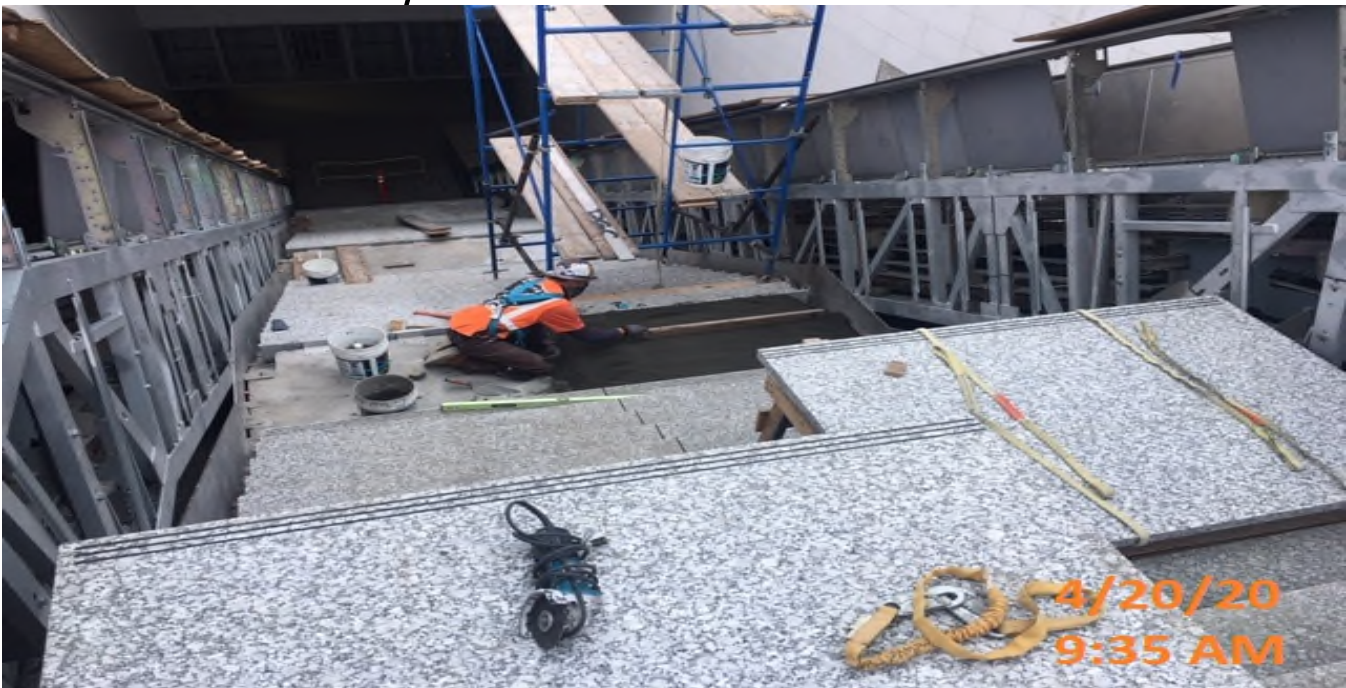
EXPO STATION – Continue granite stair tread installation at the main entrance staircase landing of the plaza level.
