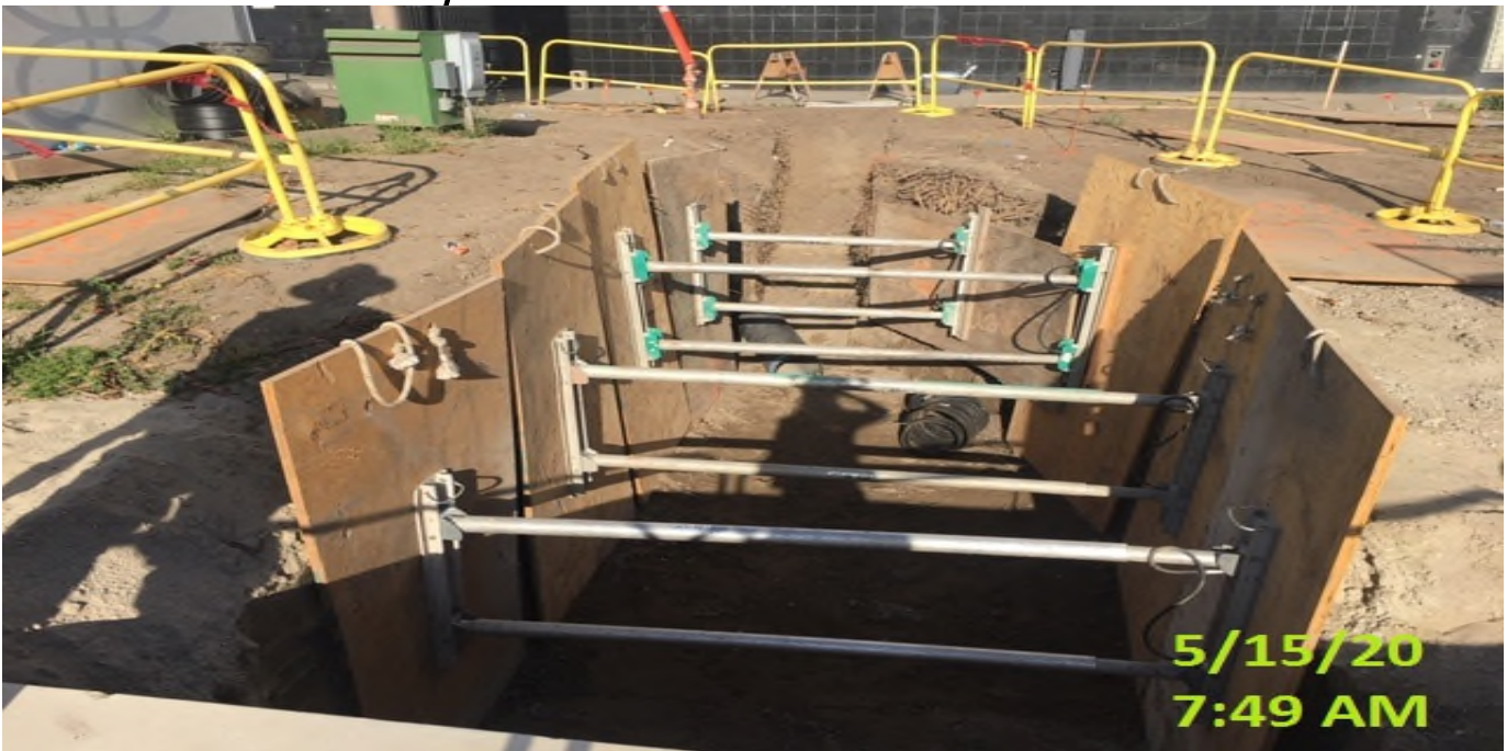
MLK STATION – Continue excavating/laying out 12” HDPE drainage pipe system connecting to Catch Basin#3 at the northern section of the plaza level.
