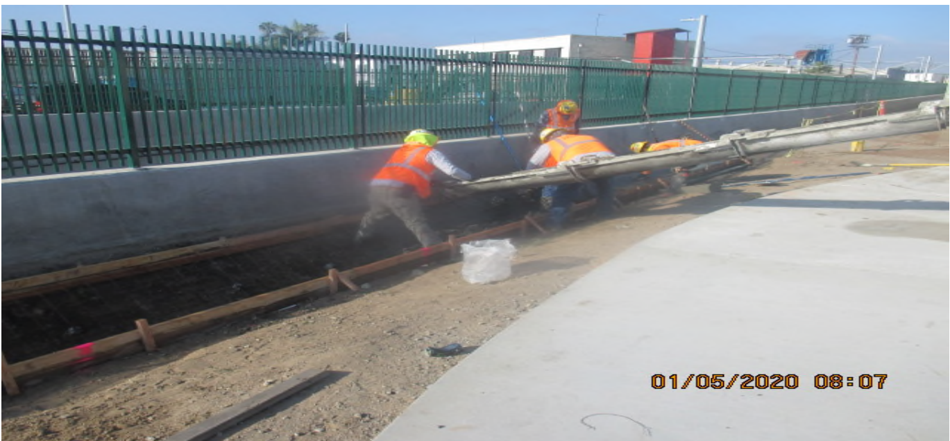
UG3 – Placing concrete for the culvert drainage system along the southbound barrier wall between Sta 278+55 – 279+25 at Victoria Yard. 5/1/20
