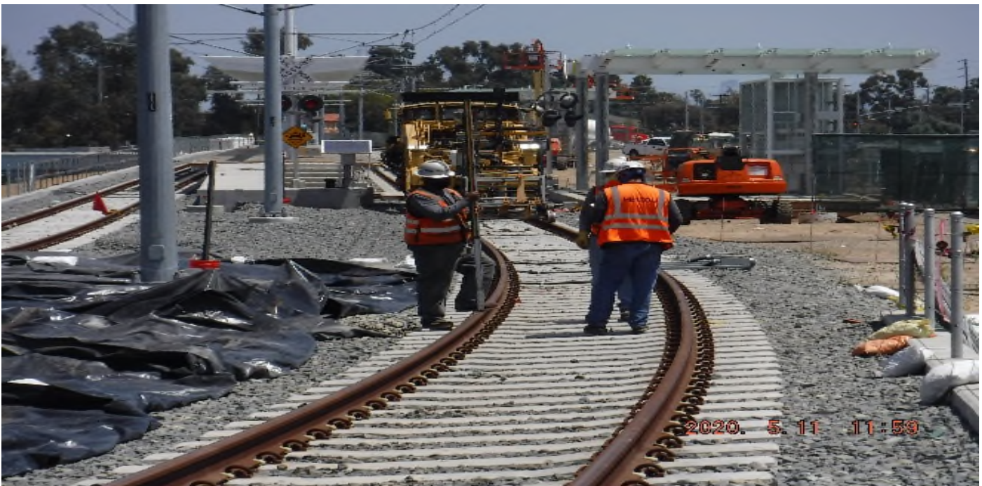
Florence/Brea - STA 205+50 TK#4,NB looking north – track geometry measurement south of La Brea Station
