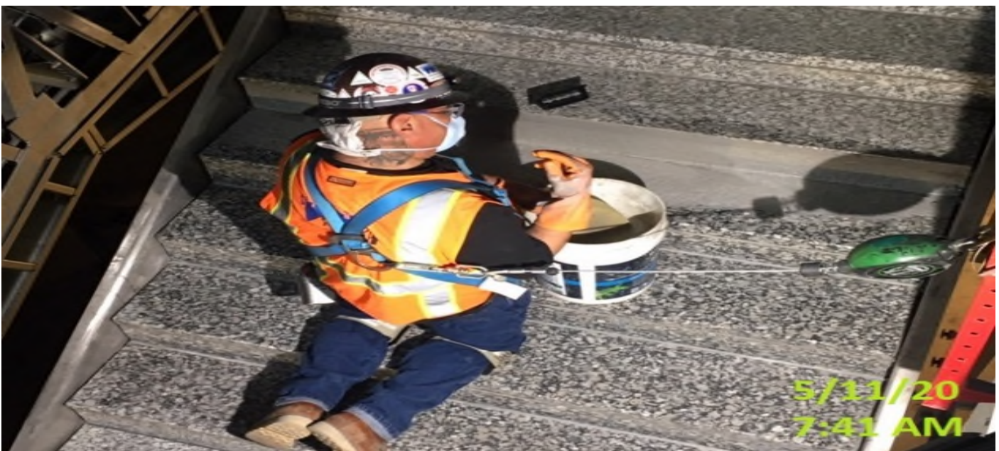
MLK STATION – Continue grouting and installing granite risers and treads for staircase 3 from concourse to platform level.
