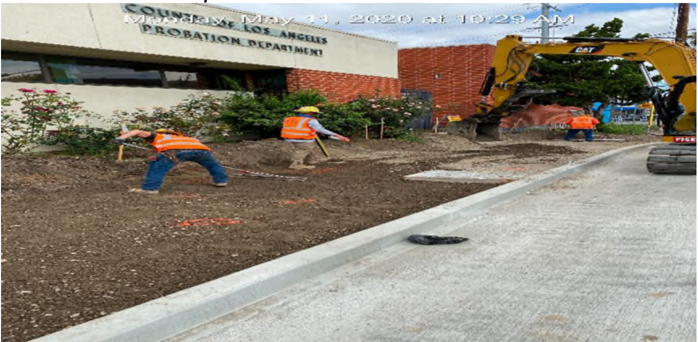
EXPO STATION – Fine grading and compacting for new sidewalk installation on southbound Crenshaw Blvd between Exposition Blvd and Rodeo Blvd.
