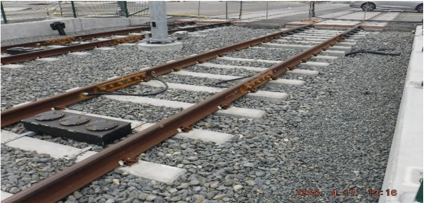
57 th Street - STA 329+75 TK#4/NB looking north – track structure status as of 4.17.2020 south of 57th St – PUNCH LIST.
