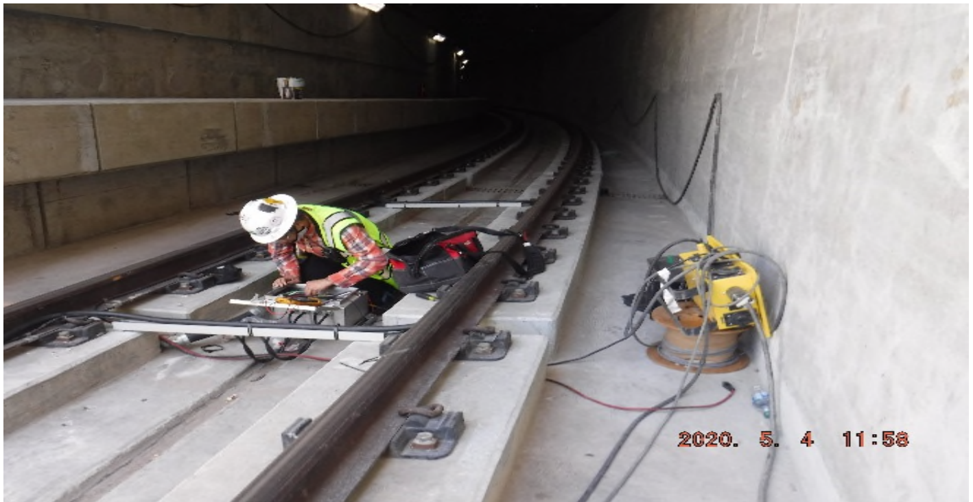
UG3 – STA 283+00 TK#4,NB looking north – TC work at south portal UG3 (Victoria).
