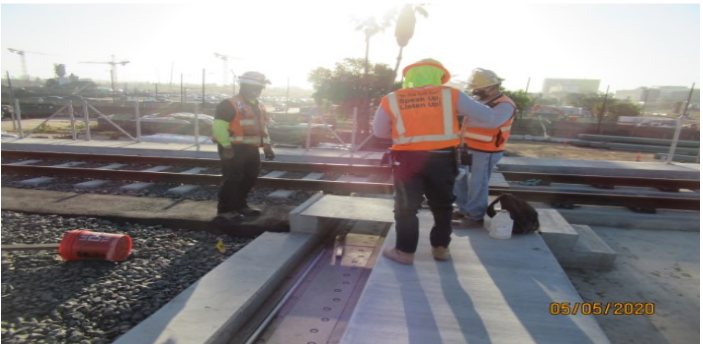
AVIATION/CENTURY - WSCC QC & concrete foreman going over open item punch list, Activity #1498 on Century/Aviation bridge (looking east)
