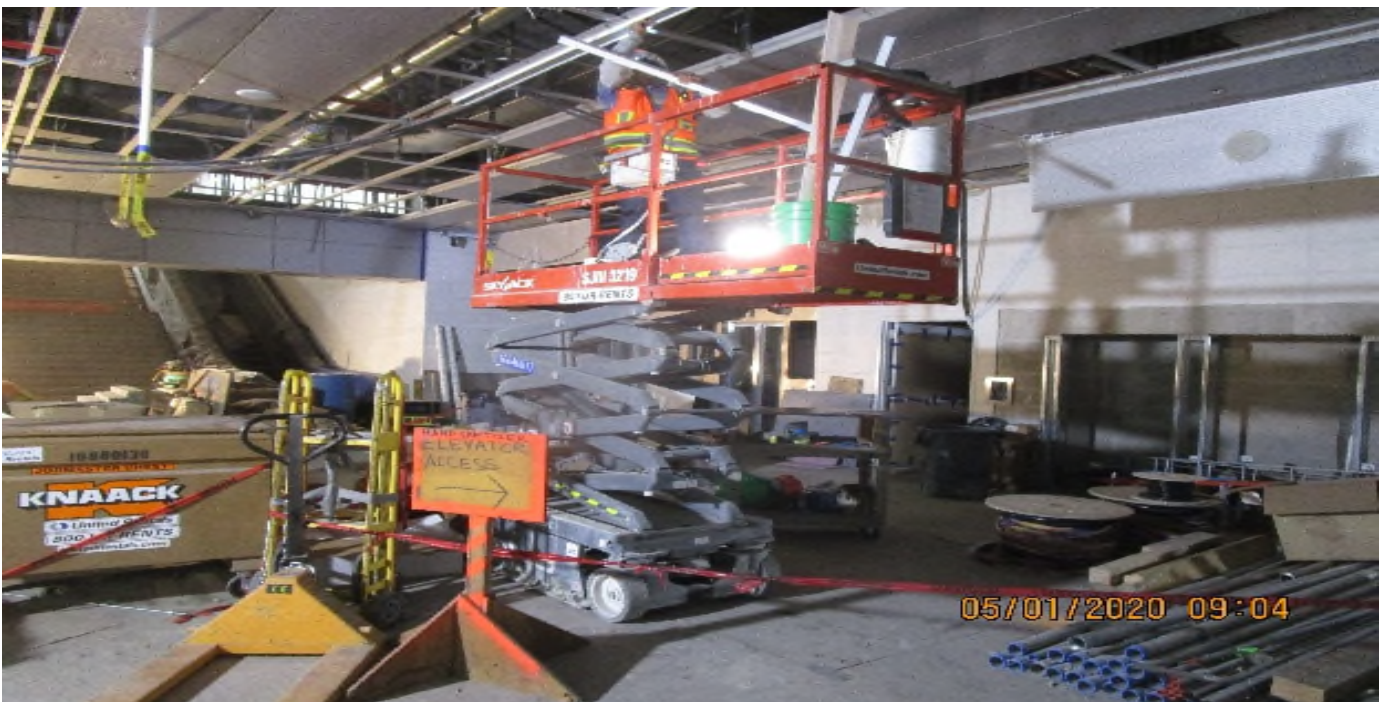
LEIMERT PARK STATION – Continue installing ceiling light fixtures at the concourse level.
