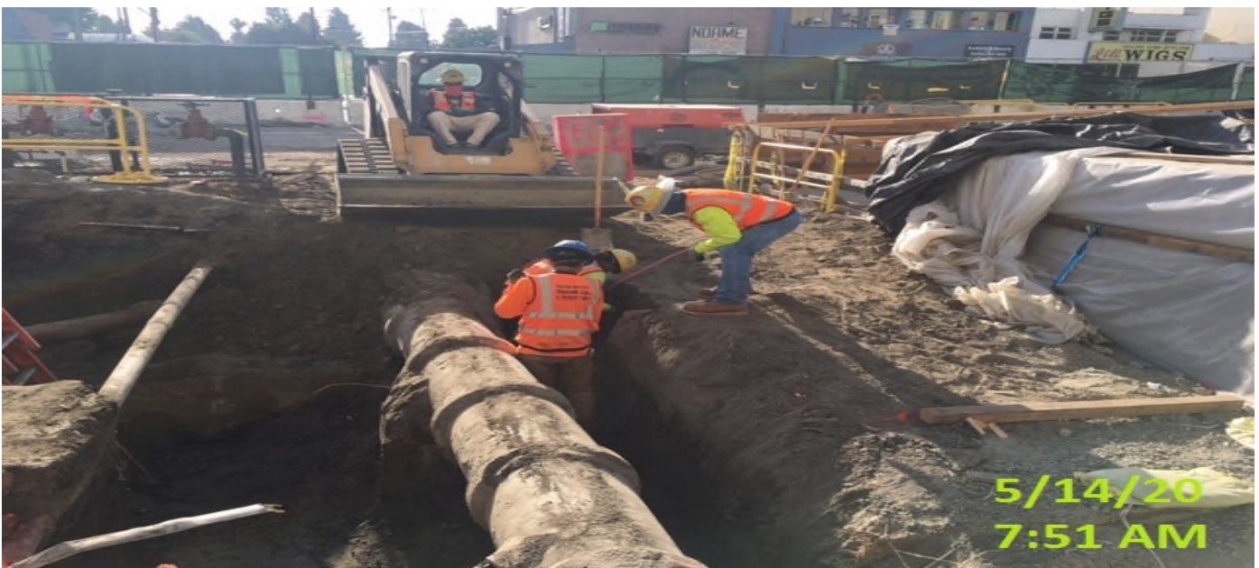
MLK STATION – Continue excavating/laying out 12” HDPE drainage pipe system at the northwest section of the plaza level.
