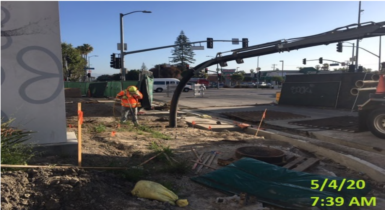
MLK STATION – Potholing and drilling to confirm placement of tree well installation at the northeast corner of the plaza.
