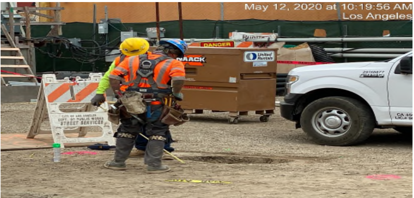
LEIMERT PARK STATION – Began layout for upcoming tree well installation at the plaza level.
