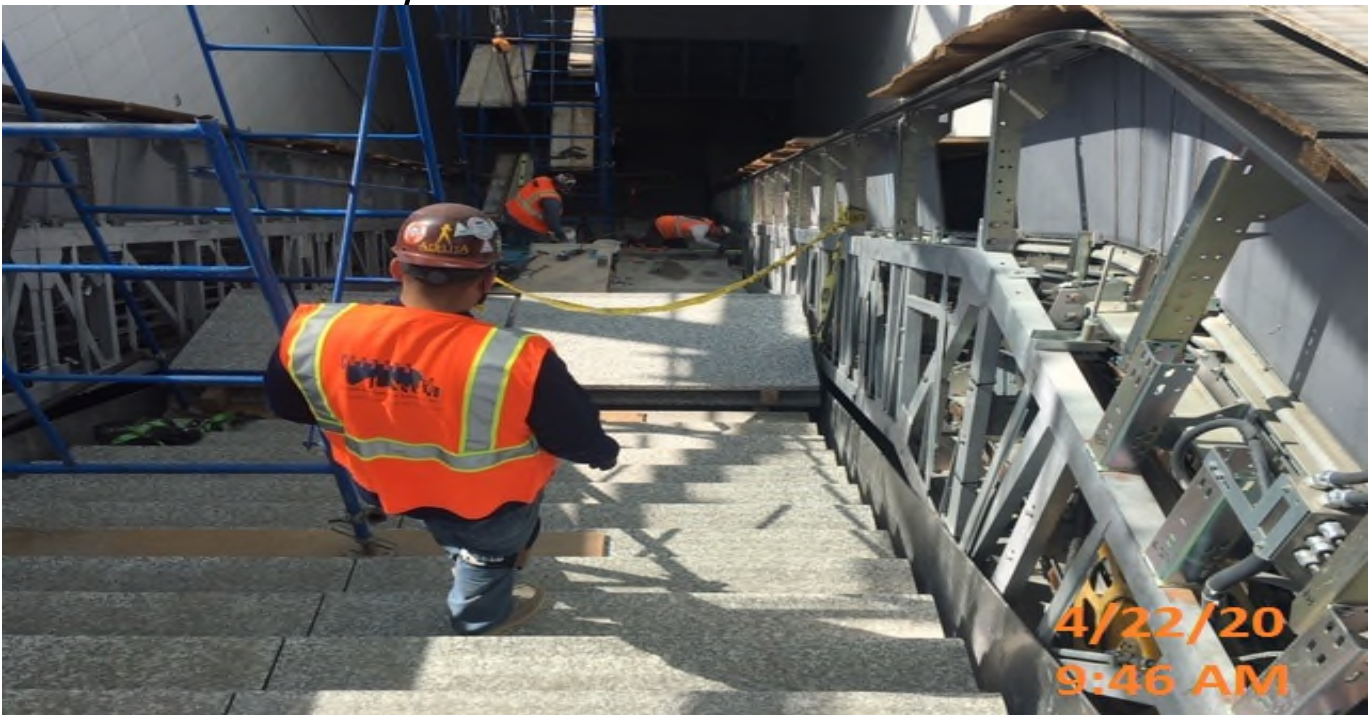
EXPO STATION – Continue granite stair landing section installation at the main entrance staircase of the plaza level.
