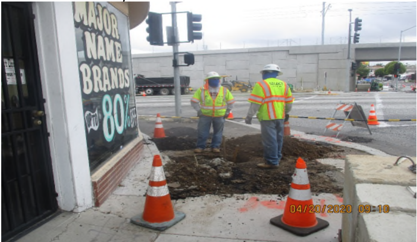
Florence/Brea – WSCC Carpenters formed for plaza platform at s-ticket pavilion La Brea Station.
