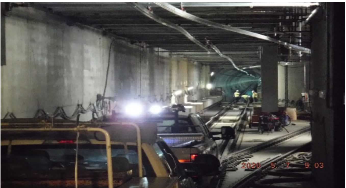
UG4 - STA 444+40 TK#4/NB looking south – system work UG4 DXO area Exposition Station.
