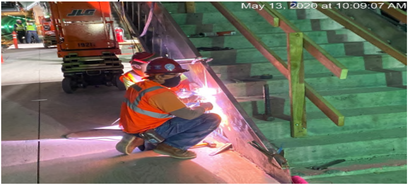
LEIMERT PARK STATION – Continue installing metal steel framing at the underside of stairwells 3&4 at the platform level.
