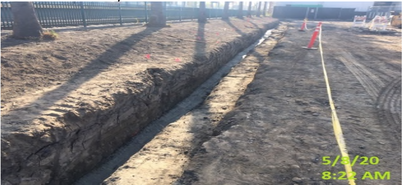
EXPO STATION – Placed concrete over the conduit duct bank along the north side section of the plaza level.
