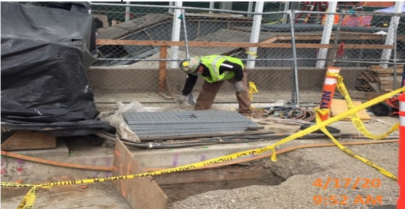
LEIMERT PARK STATION – Preparing to install catwalk frame to the main entrance canopy structure at the plaza level.
