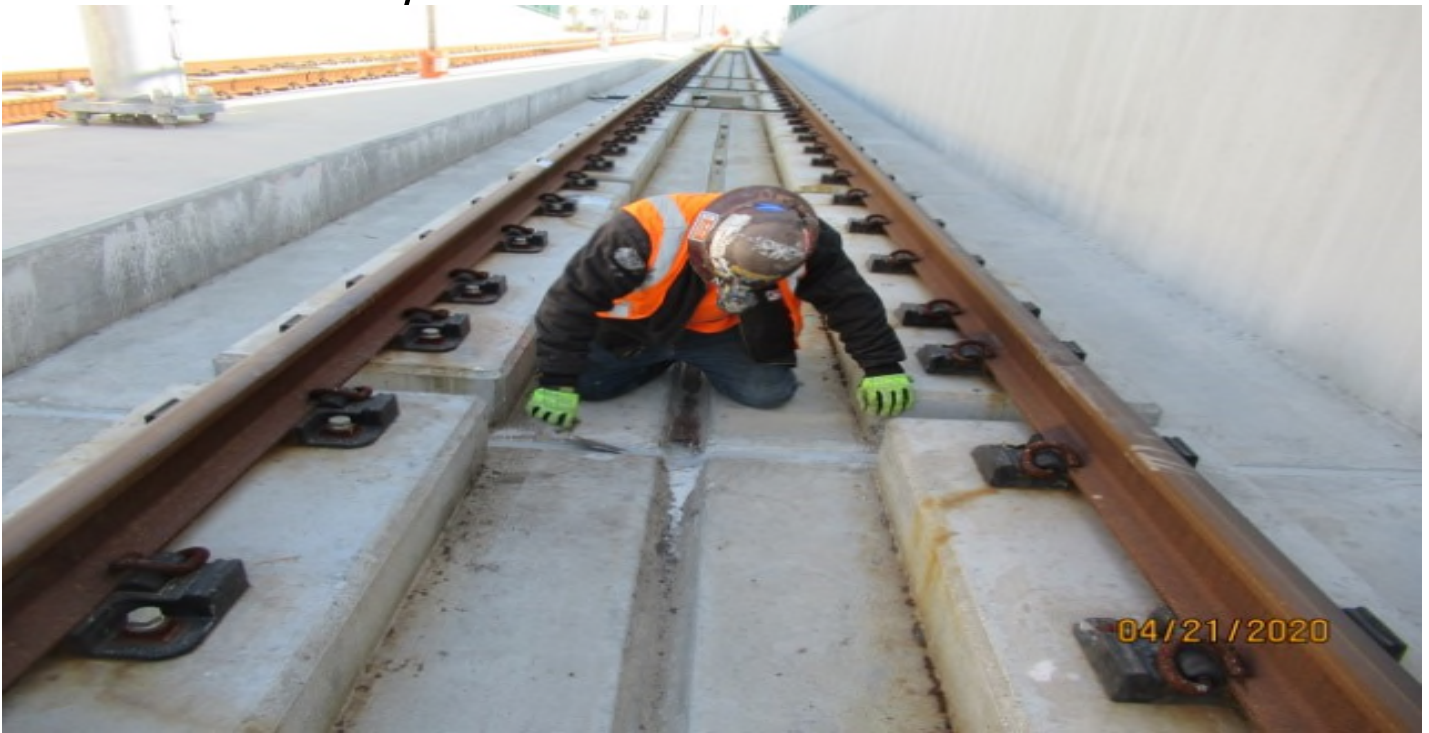
UG1 - WSCC placing epoxy on expansion joints in UG1 NB #4 track WSCC placing epoxy on expansion joints in UG1 NB #4 track out of sequence work.
