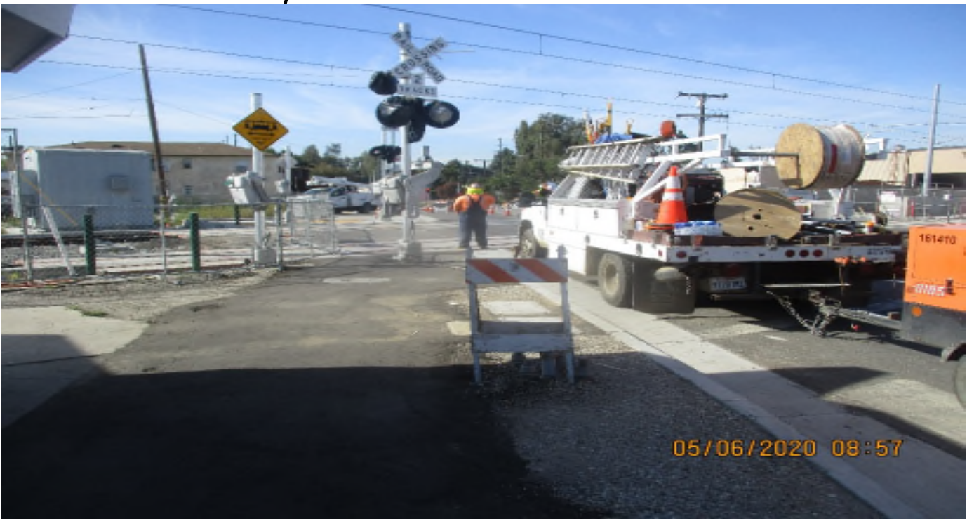
Florence/West – Select Electric Continue pulling wire and standing poles At 71St and West St.
