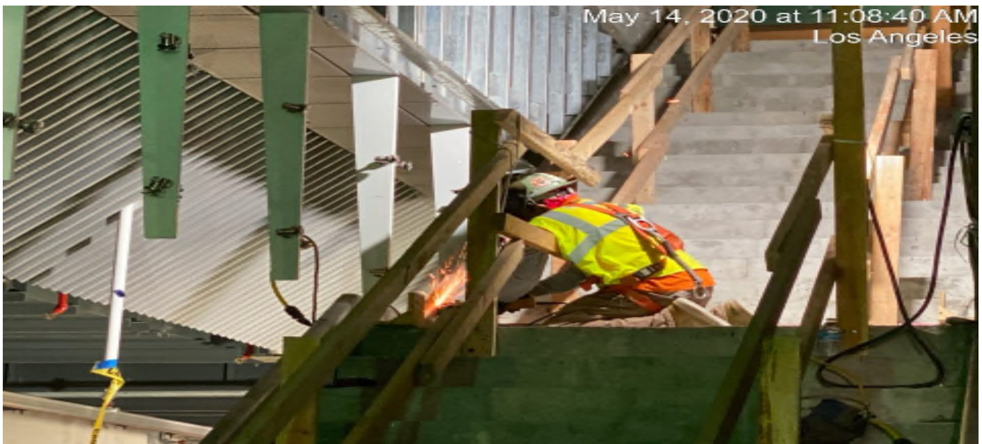
LEIMERT PARK STATION – Continue installing metal steel framing at the underside of stairwells 3&4 at the platform level.
