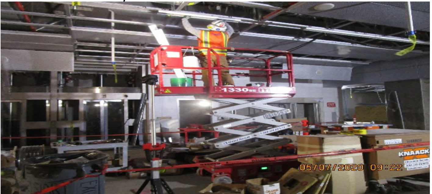
LEIMERT PARK STATION – Continue installing ceiling light fixtures at the concourse level.
