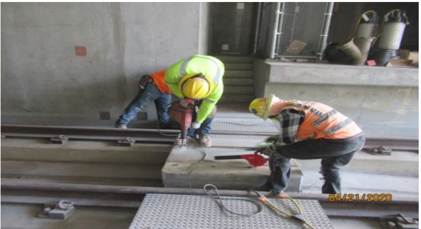
UG1 – WSCC repair work on emergency walkway crossing in UG1 SB #3 track STA 49+73
