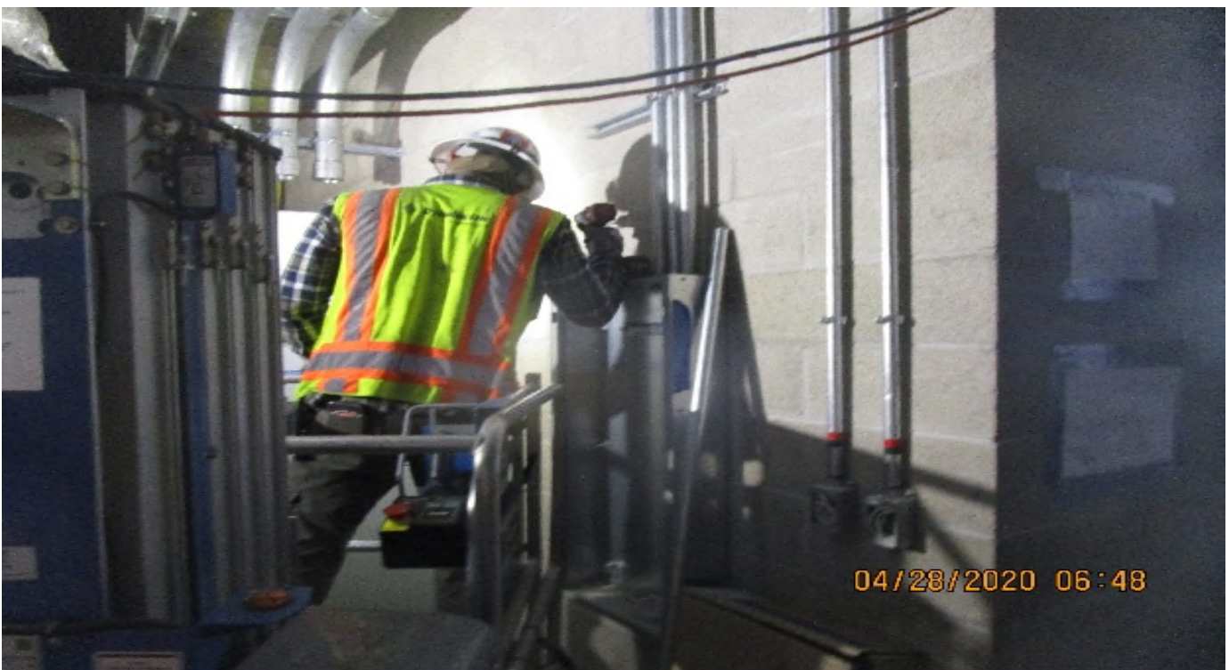
Crenshaw/Vernon - Vernon, TC&C Room C112, Resume GRC piping (3) 1" GRC from panel PP3.N to cores of Mechanical room C114.
