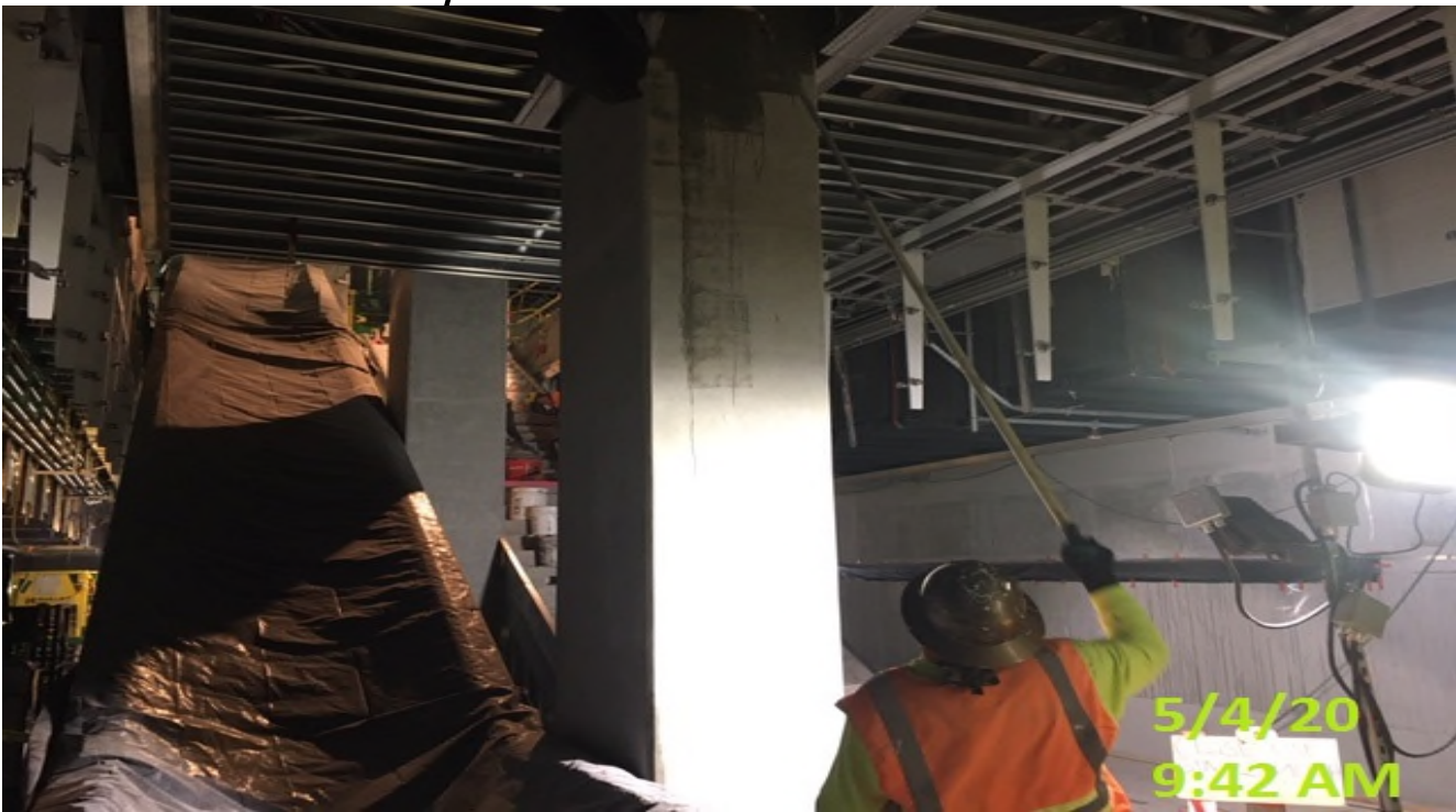
EXPO STATION – Applying anti-graffiti finish coat to all the columns at the platform level.
