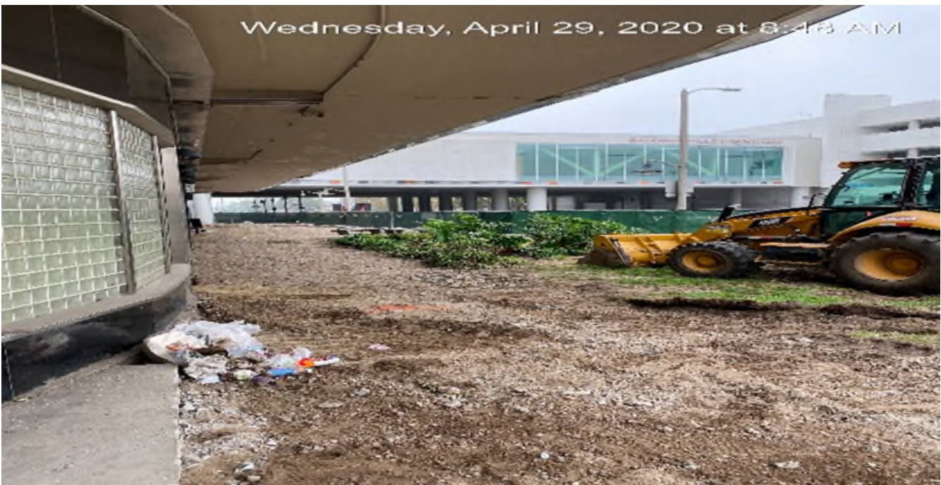
MLK STATION – Continue excavation/demolishing of the eastbound sidewalk on the northwest corner of the plaza.
