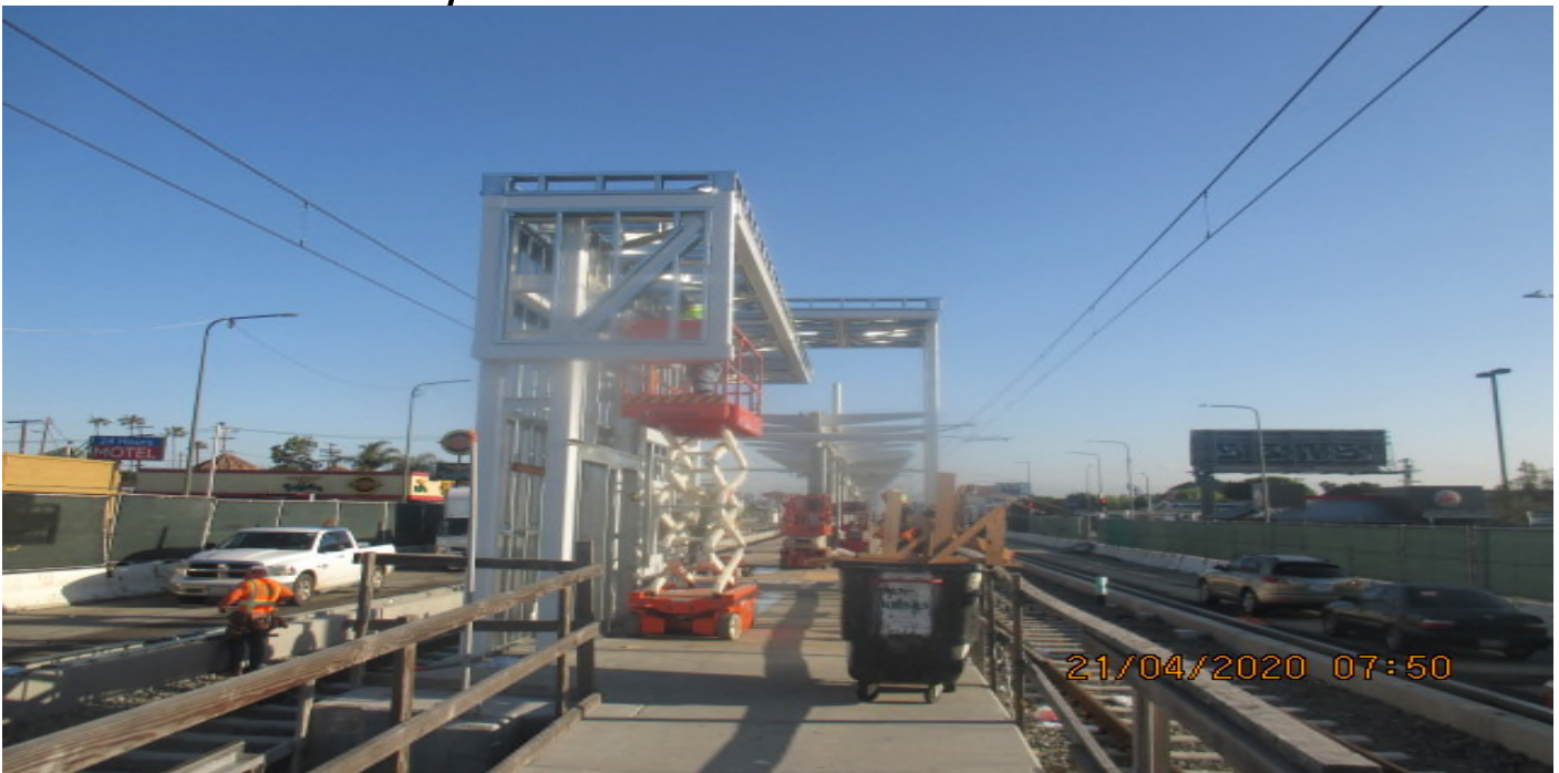
Hyde Park Station – Continue installing light gauge framing and roofing on the north and south end canopy structures. 4/21/20
