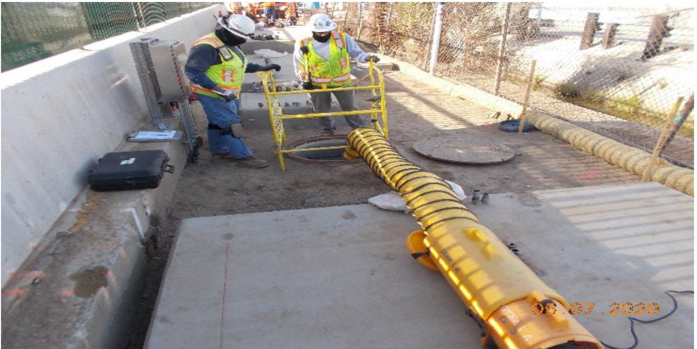
104 th Street - South view of Aux Power manhole and Dyna Electric. 104 th
