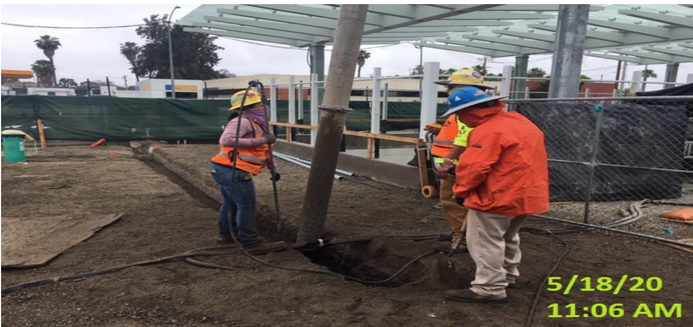
EXPO STATION – Continue trenching/potholing for conduit duct bank installation at the plaza level.
