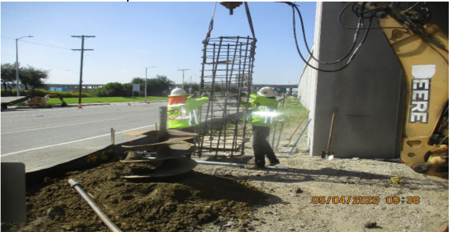
AVIATION/CENTURY - DB Electrical Place cage for SL at S/W corner of Aviation and 111th.
