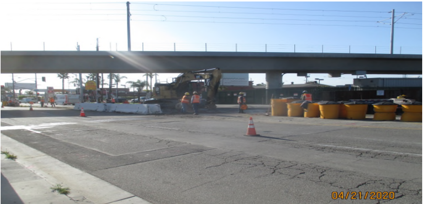
Manchester Bridge – Moving K rail and clean up to start the demo at Manchester.
