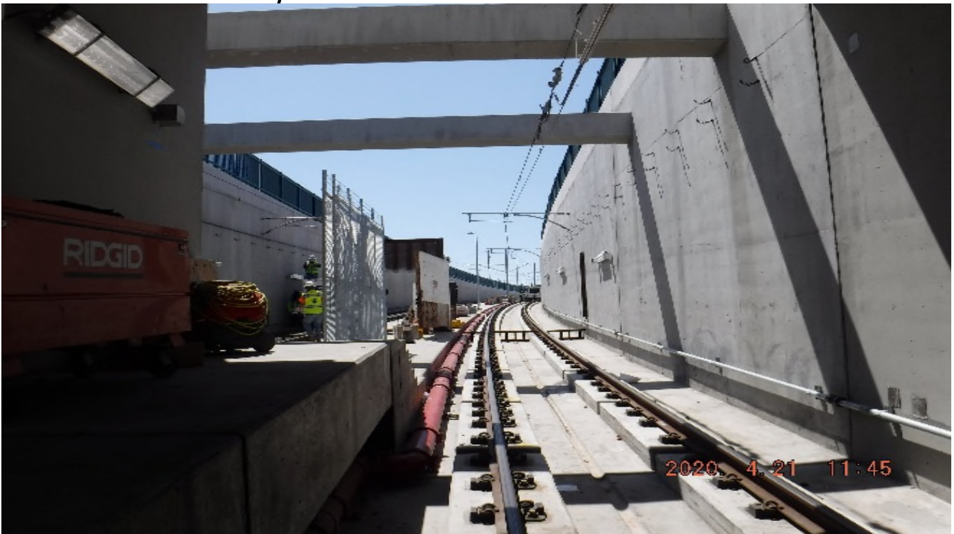
UG-4- STA 371+00 TK#3/SB looking south – OCS work south portal UG4 (48th St).
