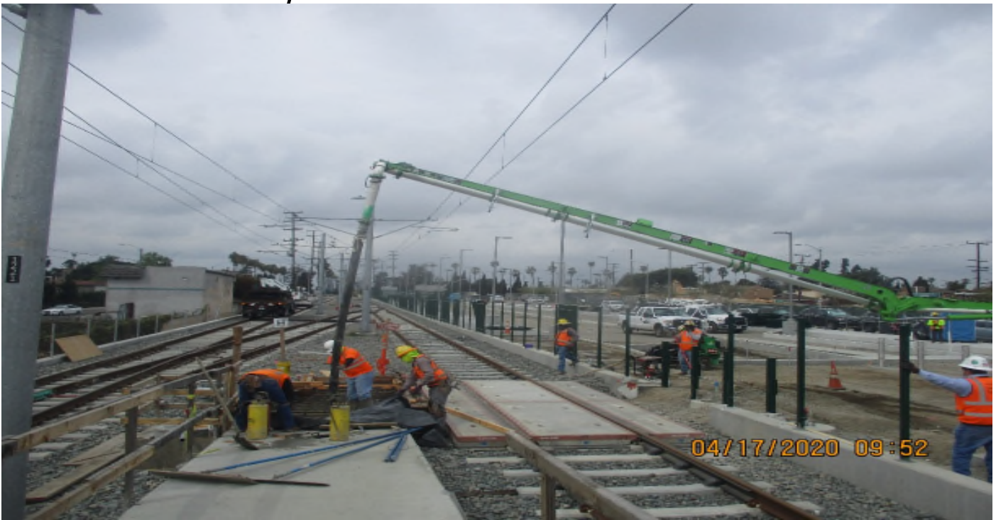
Florence/West – WSCC Placed concrete for handy capped ramp on West end of West Station.
