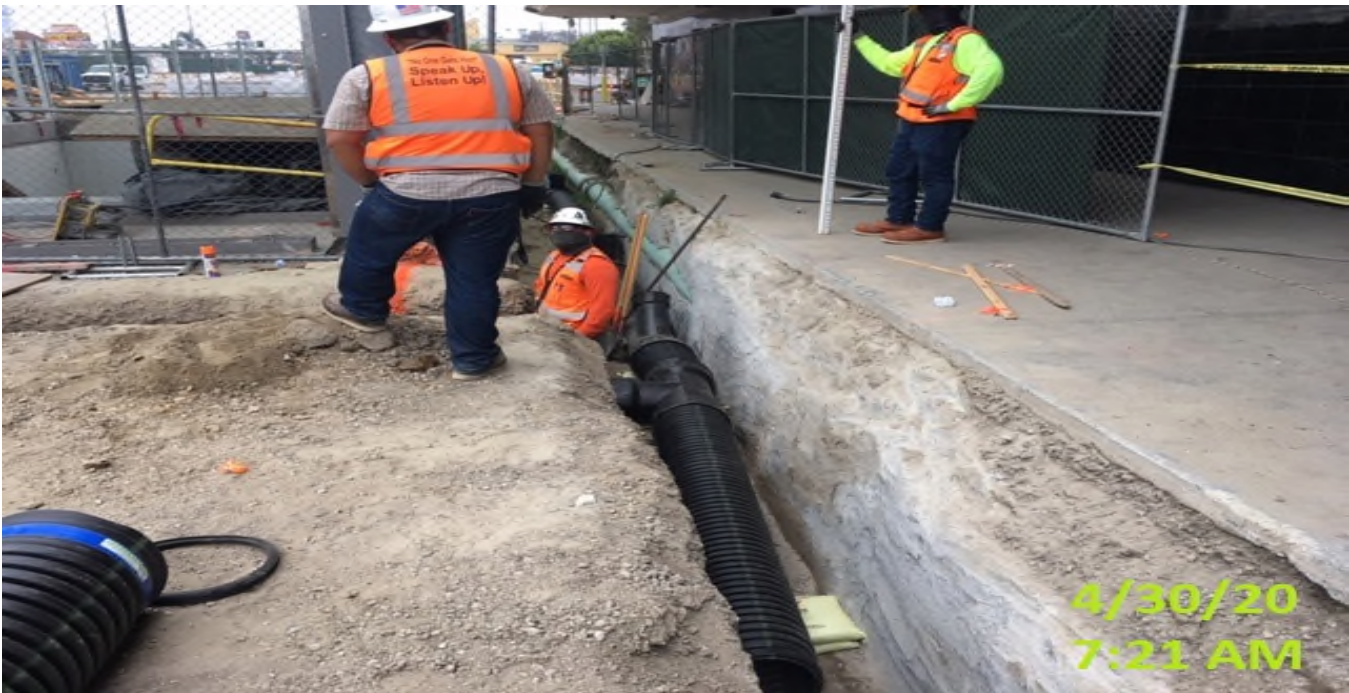
MLK STATION – Continue installing 12” HDPE drainage pipe on the west side of the plaza level.
