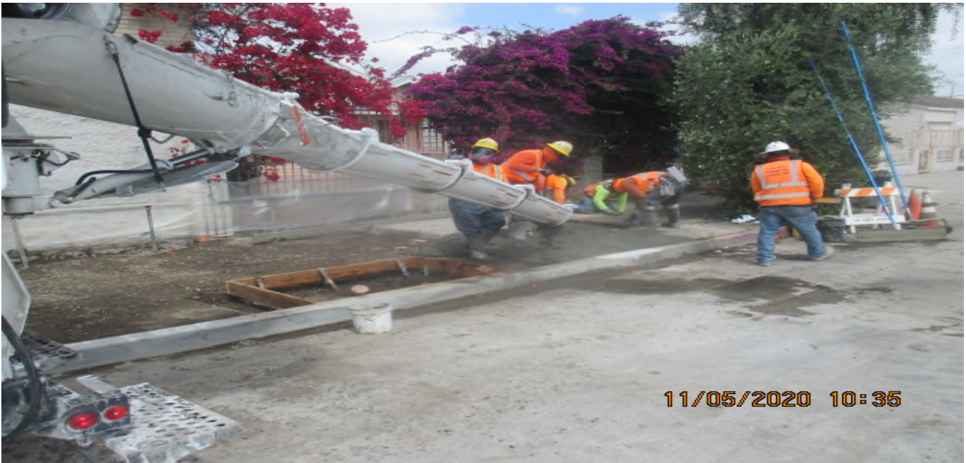
UG3 – Installing block out forms for tree wells and placing concrete for sidewalk panels at the east section of Victoria Yard. 5/11/20
