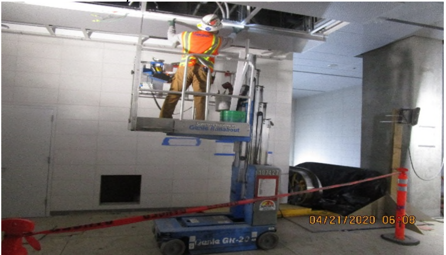
Crenshaw/Vernon - Vernon Concourse, Paid Area C146, continued rough in of AL1A-Lumium brand lighting fixtures at light pockets
