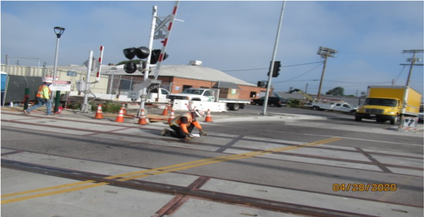
HINDRY STATION- WSCC Qc inspector verifying cross level on SB #3 track at Hindry grade crossing for BIM360 internal punch list updates (looking west)
