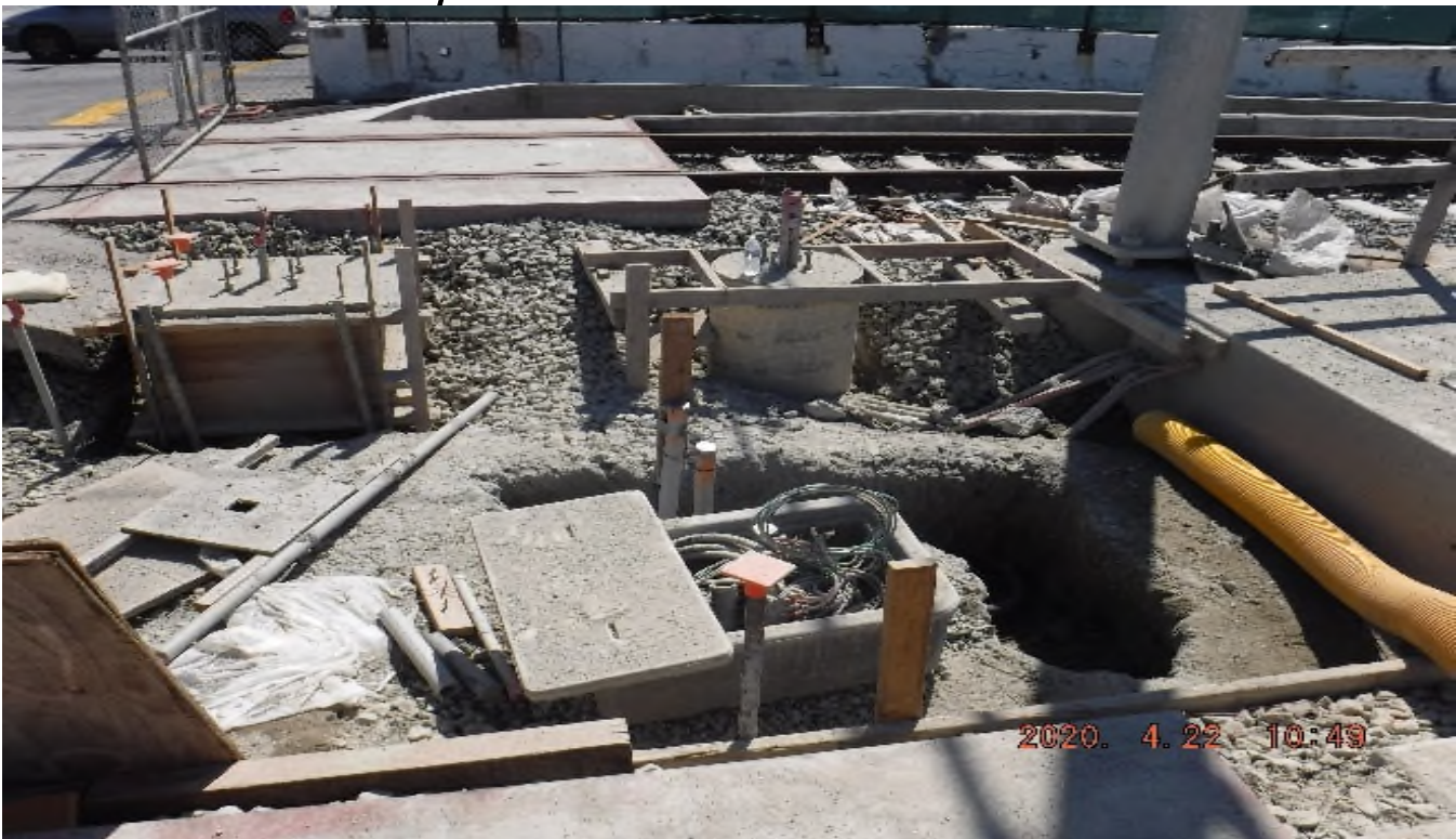
Crenshaw / Slauson - STA 323+00 TK#3/SB looking west – track structure disturbed (between tracks) north end of Slauson Station – PUNCH LIST
