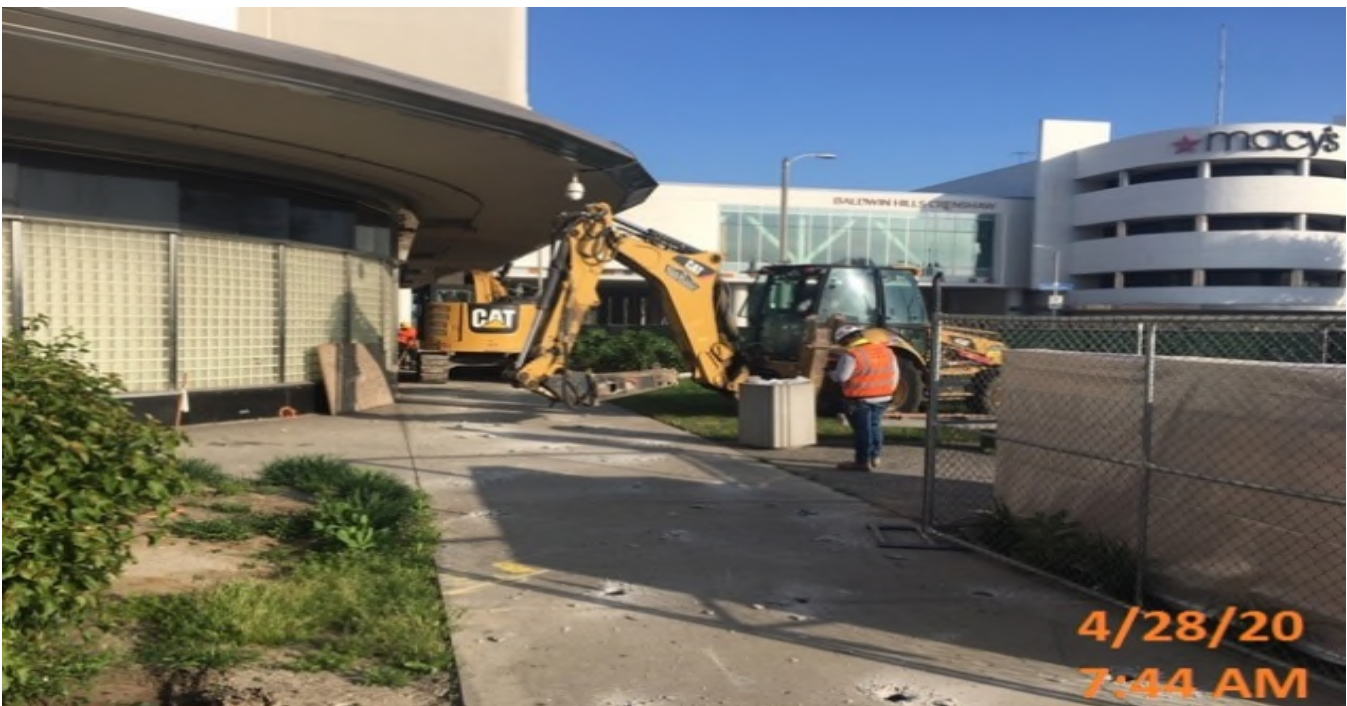
MLK STATION – Continue excavation/demolishing of the eastbound sidewalk on the northwest corner of the plaza.
