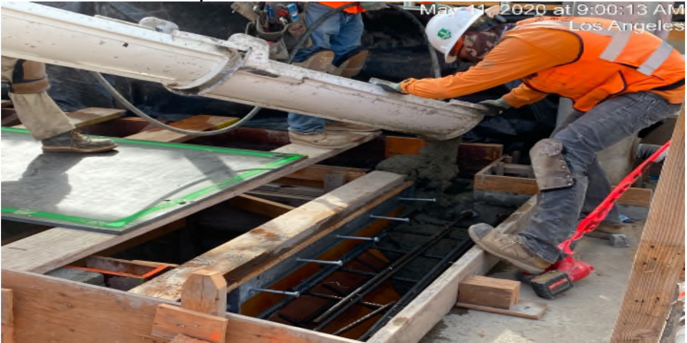
LEIMERT PARK STATION – Placing concrete for the north emergency exit hatch doors at the plaza level.
