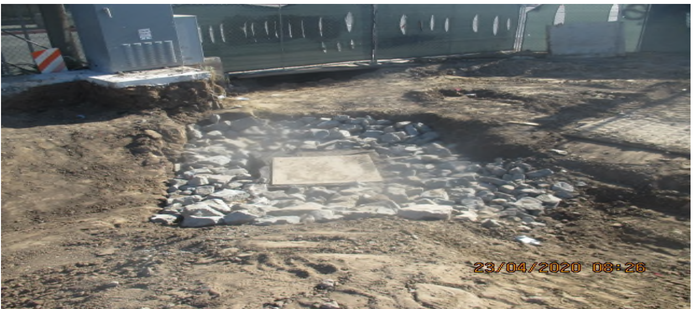
UG3 – Completed stone installation for the culvert swale drainage intersection on the north east corner of Victoria Yard. 4/23/20
