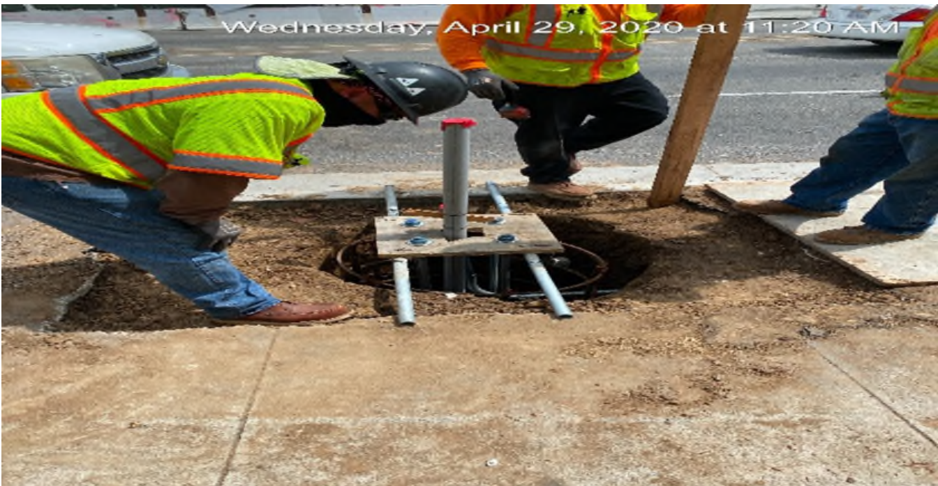
LEIMERT PARK STATION – Continue light pole foundation installation on the northeast corner of 43rd Pl and Crenshaw Blvd.
