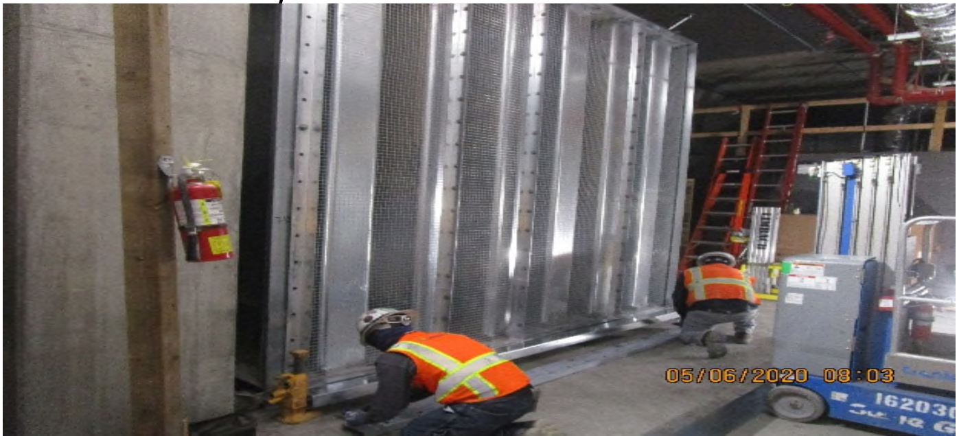
MLK STATION – Continue hardware support installation for TFD-7-122 in the North Emergency Fan Room C – 142 of the concourse level.
