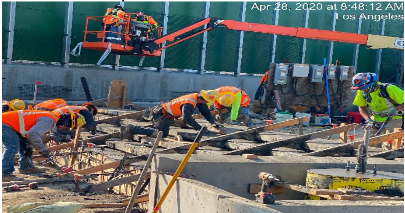
LEIMERT PARK STATION – Placed concrete and continue formwork for the planter stair risers on the northwest section of the plaza level.
