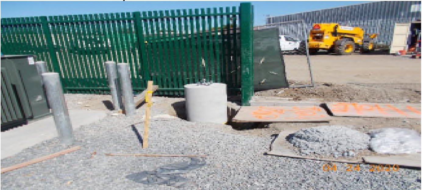
UG3 – Completed light pole foundations on both sides of the Auxiliary Power Bungalow at Victoria Yard.
