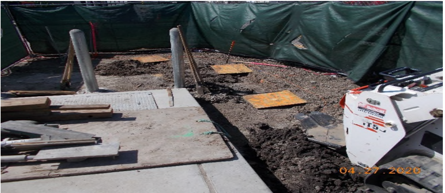
PARK MESA – Began fence post installation around the perimeter of TPSS#7 on 60th St & Crenshaw Blvd.
