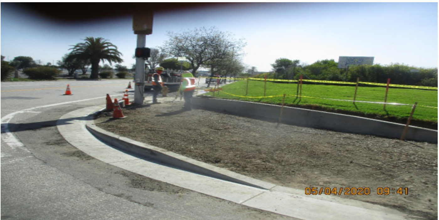
AVIATION/CENTURY - WSCC Cut SWK grade at S/E COR of 111th and Aviation
