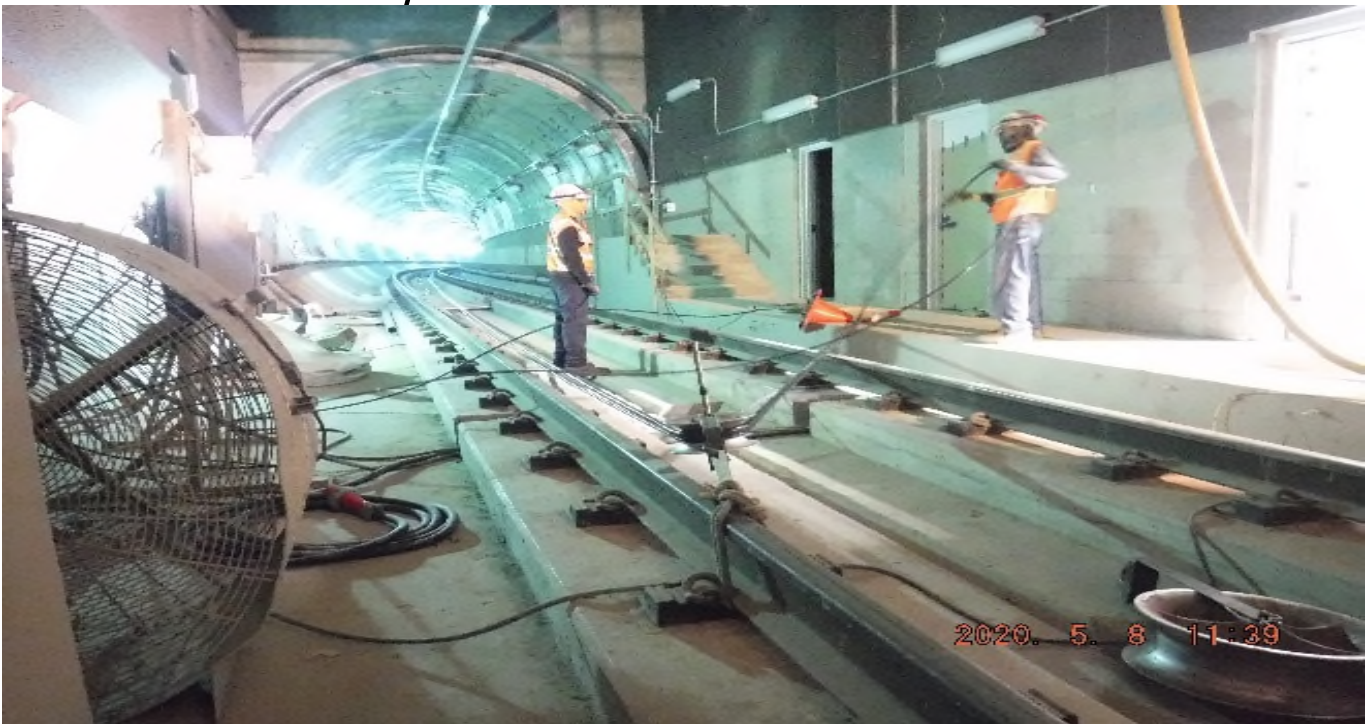
UG4 - STA 383+00 TK#3/SB looking north – set cables in duct bank UG4 Vernon Station north.
