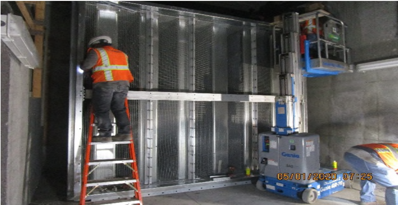
MLK STATION – Continue hardware support installation to TFD-7-322 in the North Tunnel Vent Plenum C – 140 of the concourse level.
