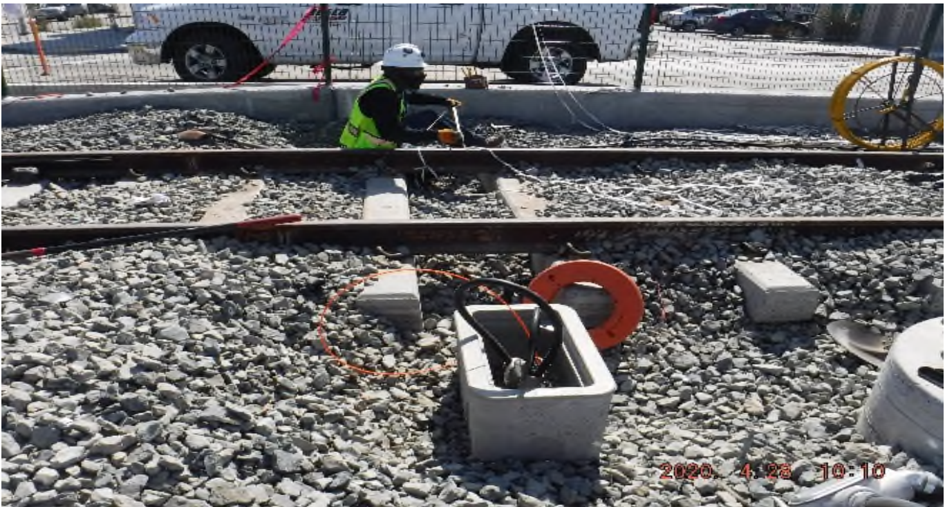
57th STREET- STA 329+90 TK#4 , NB looking east – system work with track structure disturbance south of 57th St – PUNCH LIST
