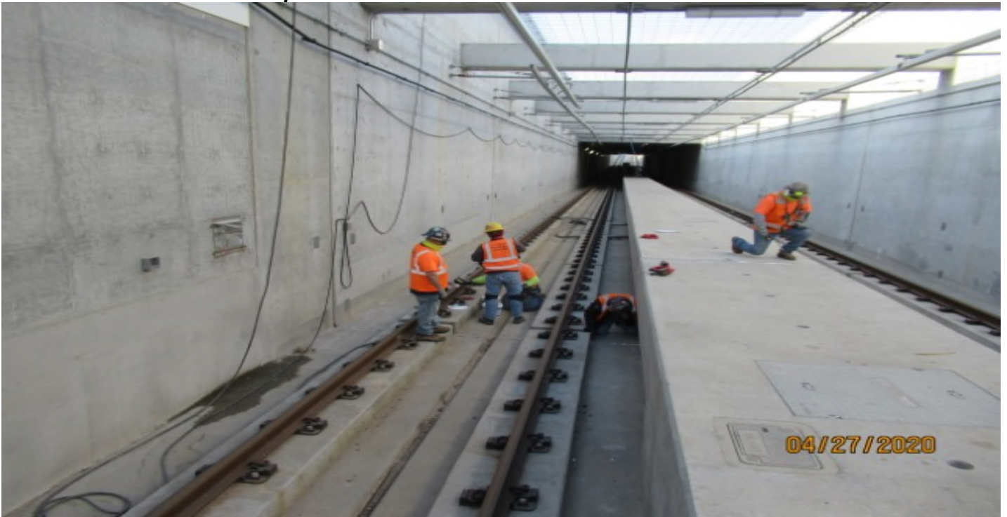
UG1- WSCC installing epoxy into expansion joints in UG1 NB #4 track (looking south) out of sequence
