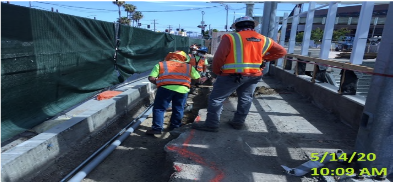
EXPO STATION – Continue trenching for conduit duct bank installation at the southwest corner of the plaza level.
