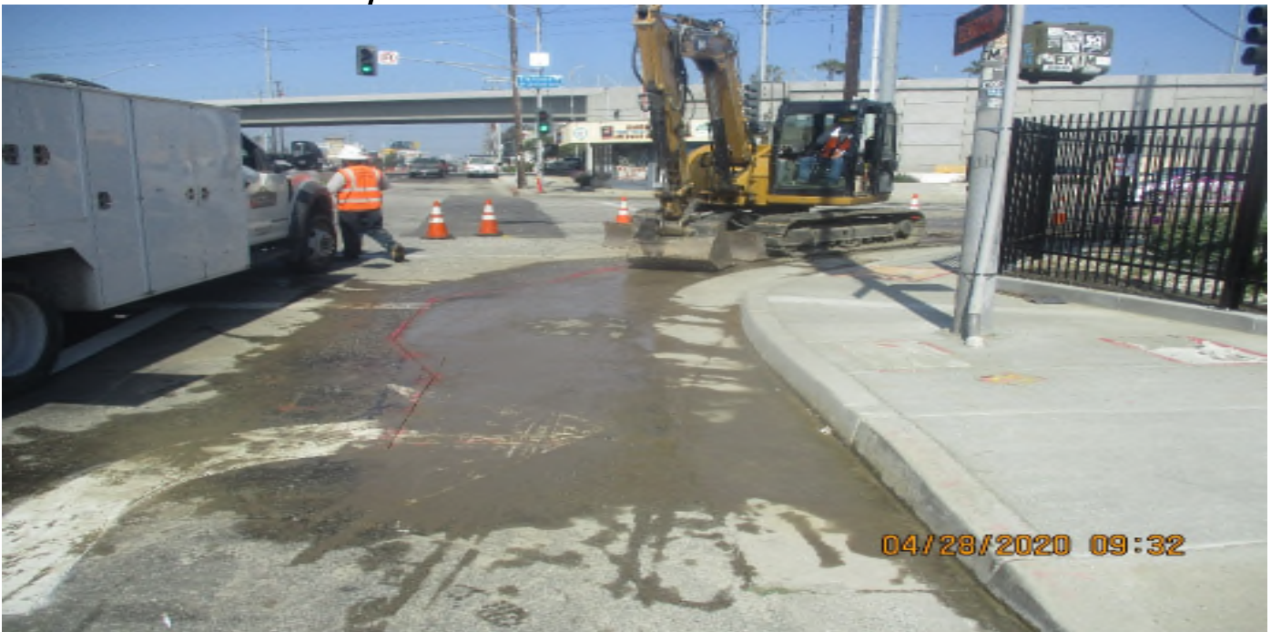
MANCHESTER STREET- WSCC Saw cut and remove street at N,E COR of Manchester and Florence.
