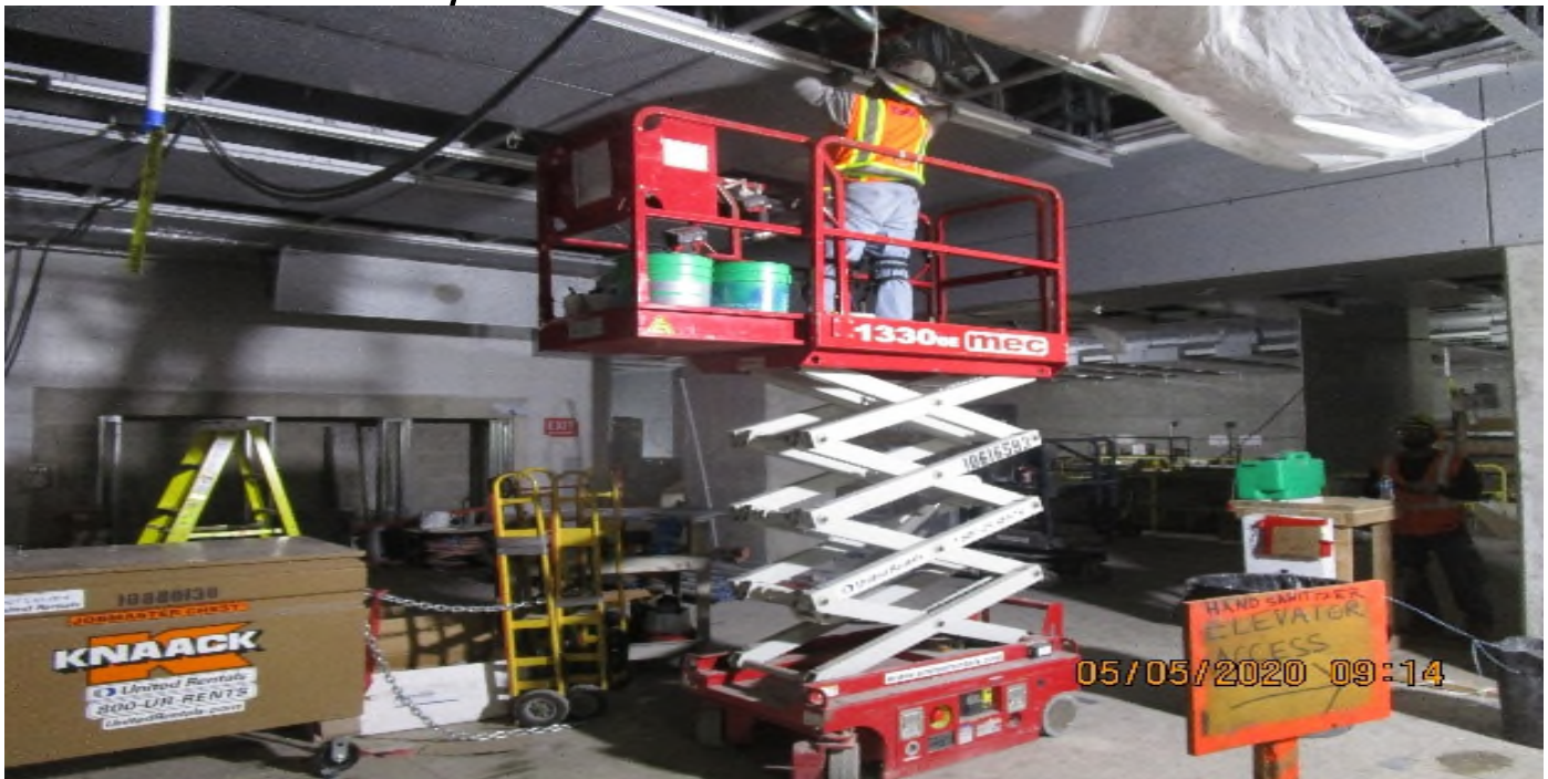
LEIMERT PARK STATION – Continue installing ceiling light fixtures at the concourse level.
