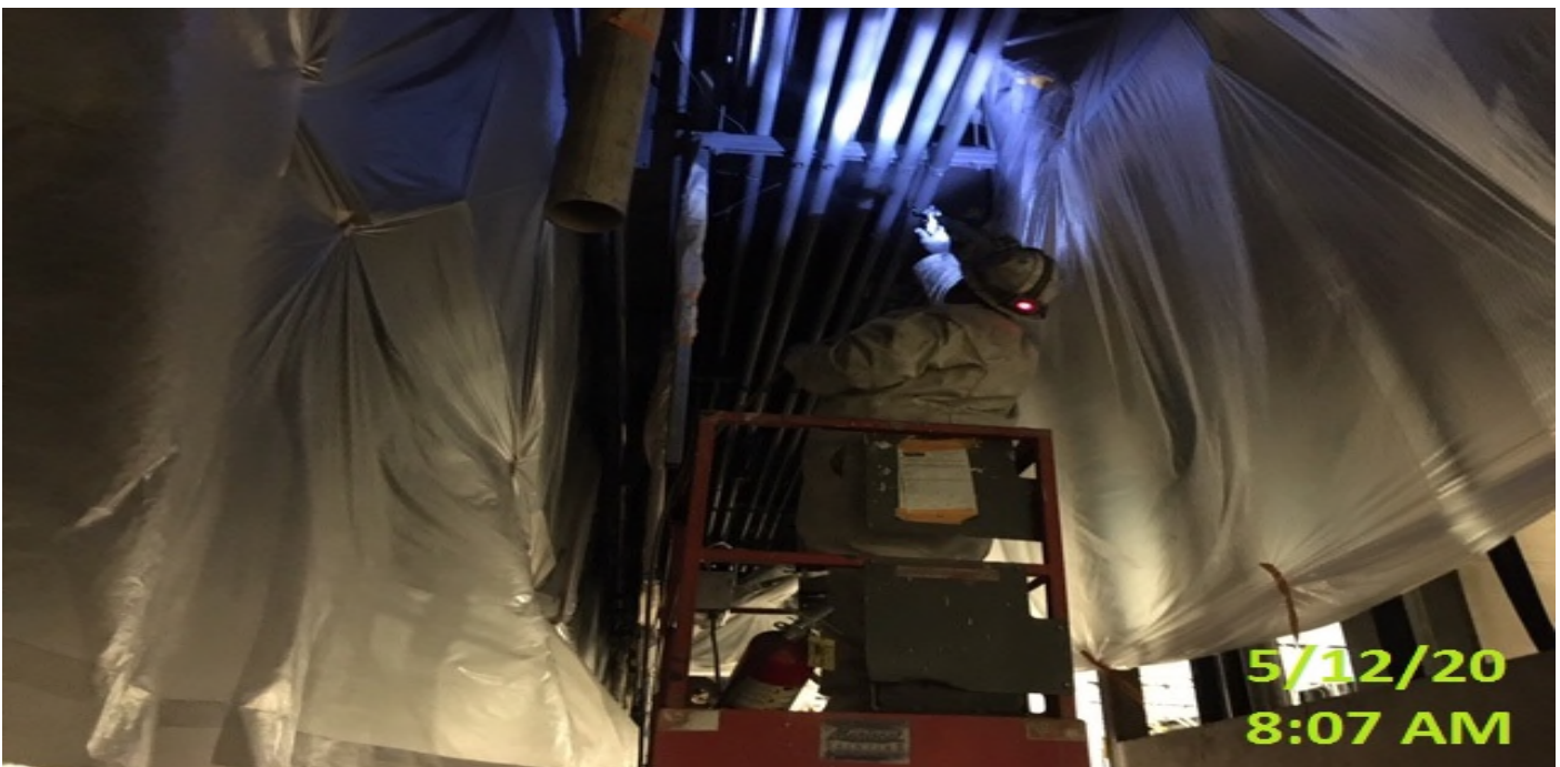
MLK STATION – Applying finish paint to the ceiling conduits at the platform level.
