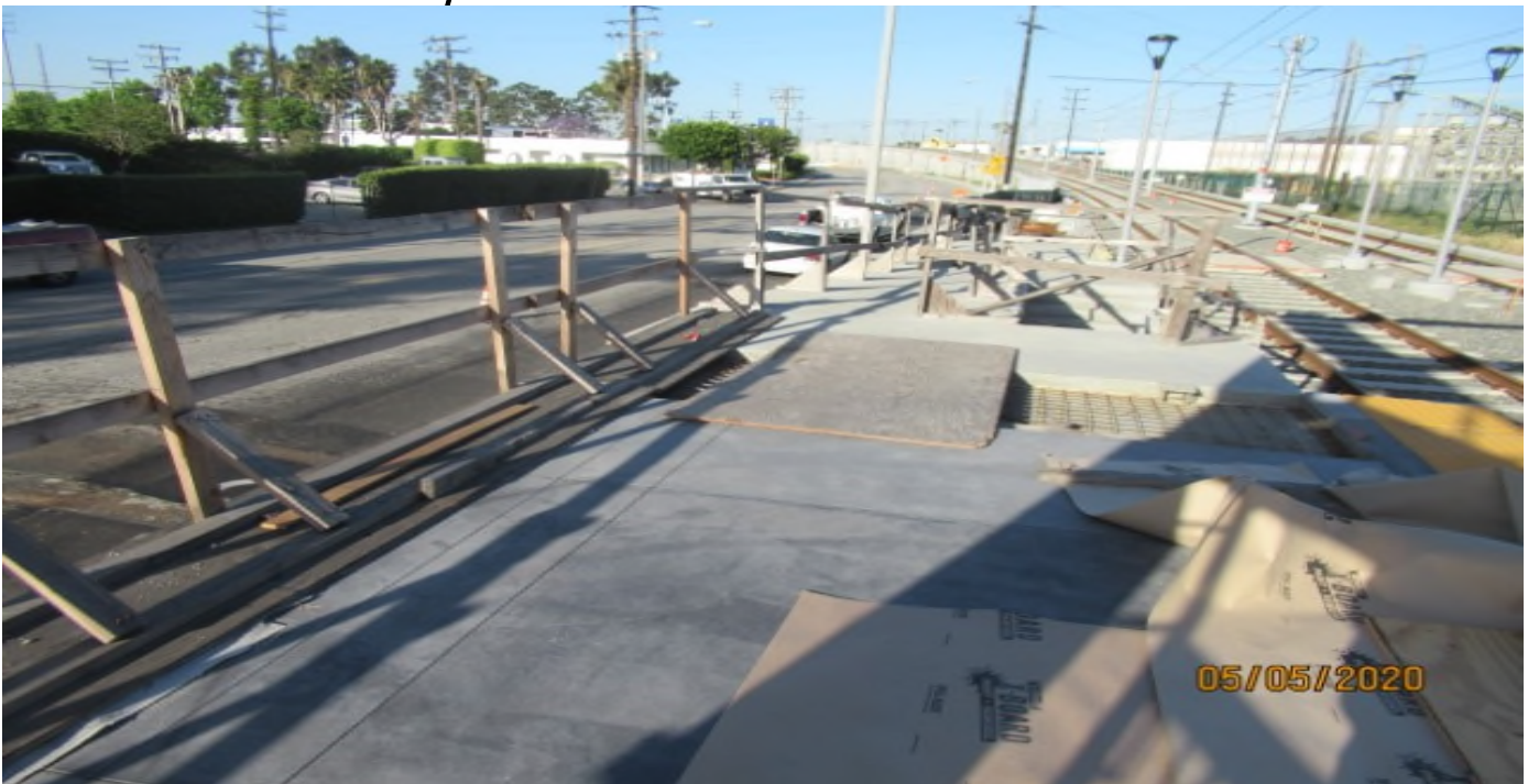
HINDRY STATION- Hindry Station platform #4 NB track, being covered with plywood sheets (looking south)
