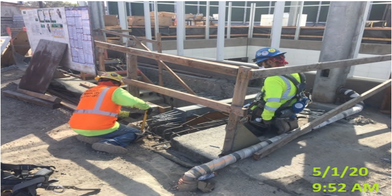
LEIMERT PARK STATION – Installing steel framing for the north emergency exit hatch doors at the plaza level.
