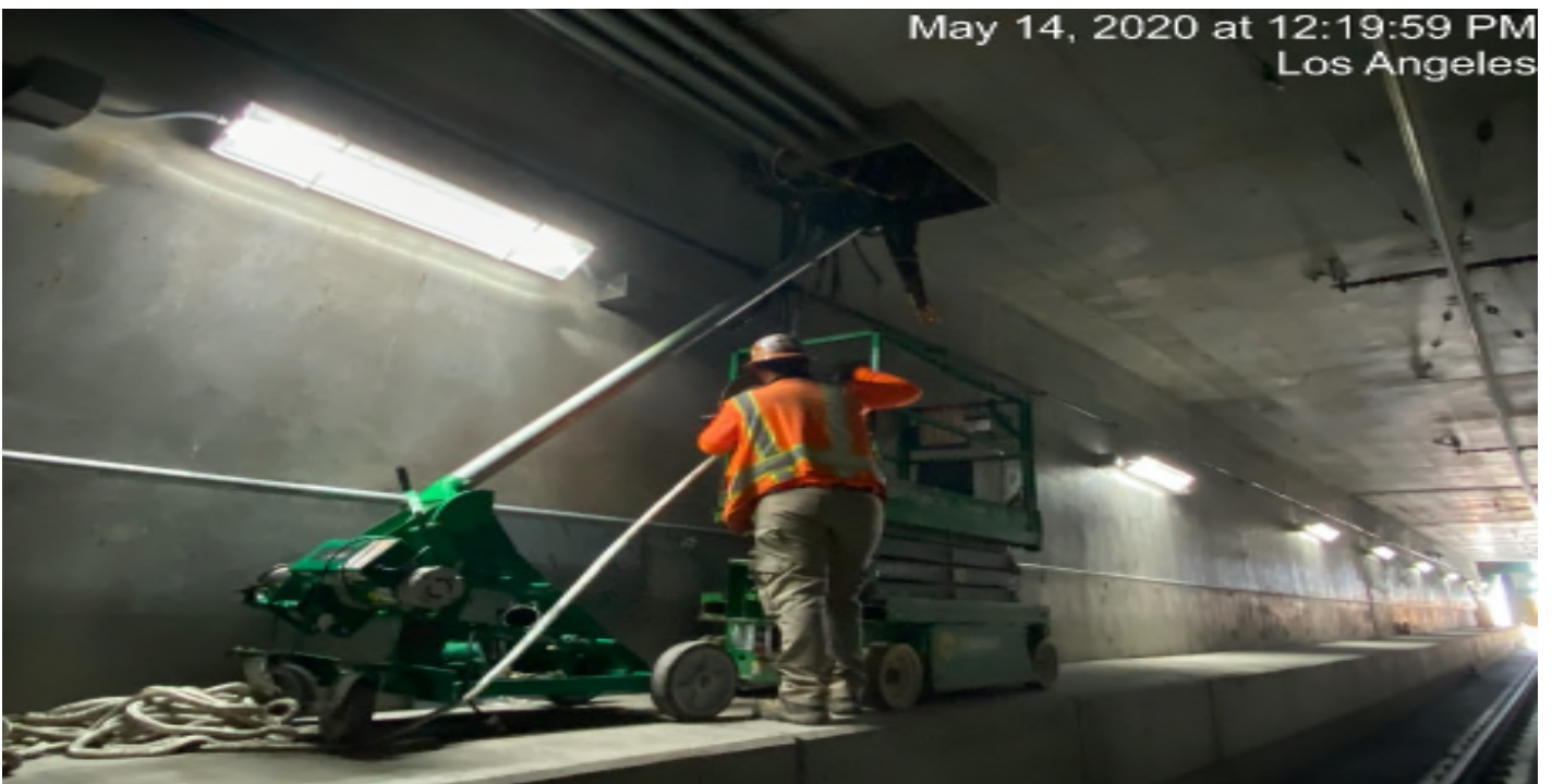
UG3 – Continue pulling permanent power cables for the tunnel booster fans along the northbound tunnel.
