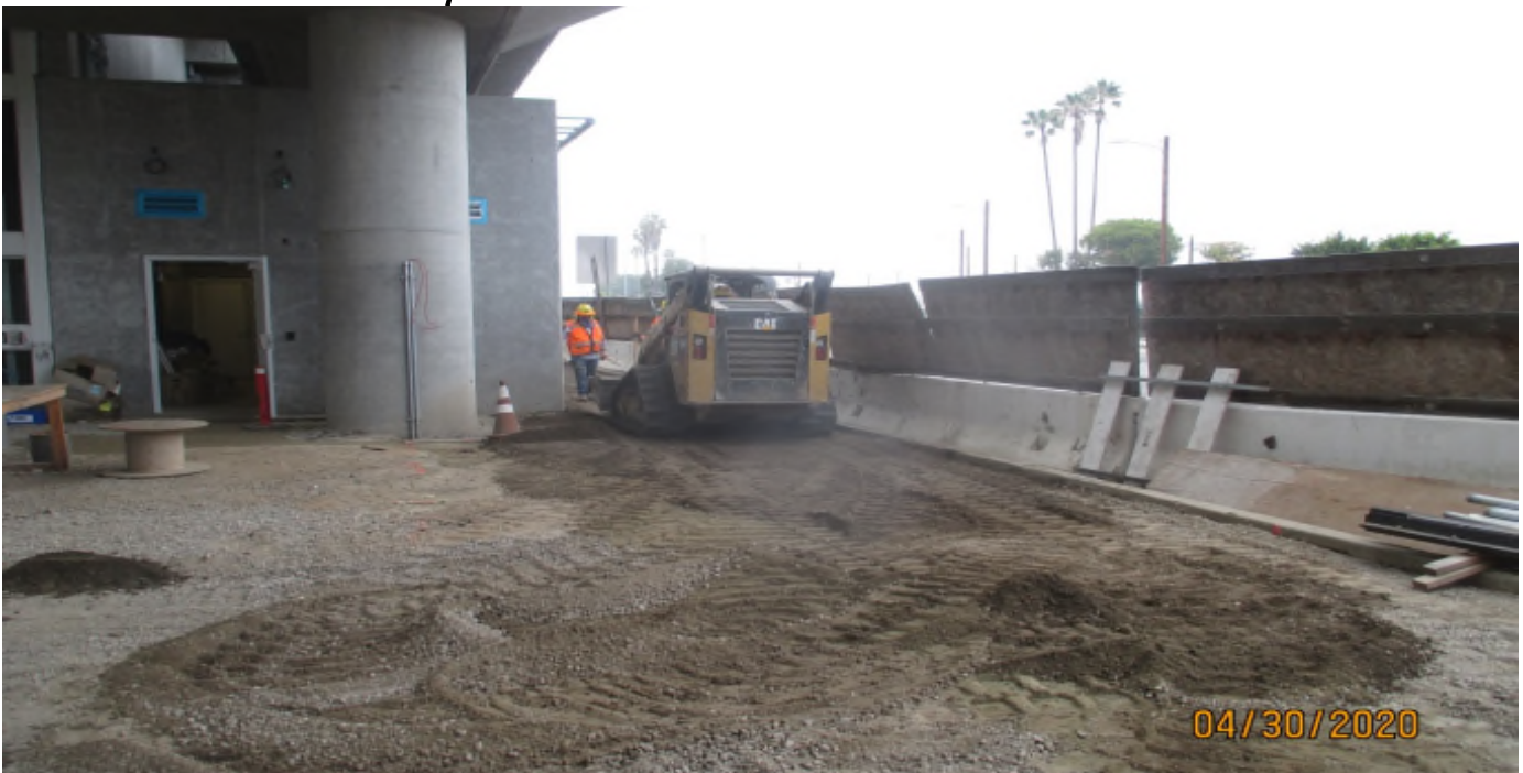
Aviation/Century – Placing base on the east side of the Aviation Station service building.
