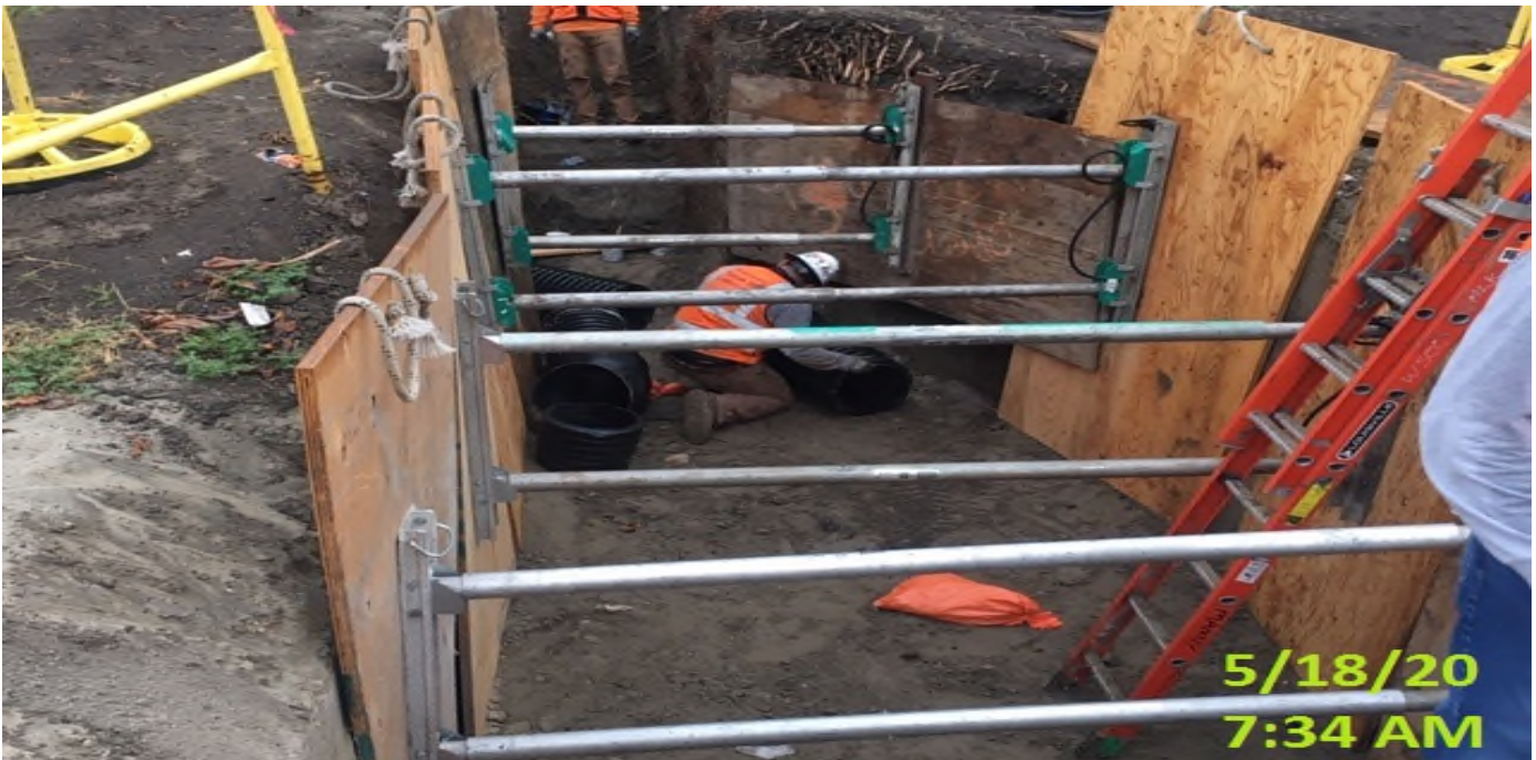
MLK STATION – Continue laying out 12” HDPE drainage pipe system connecting to Catch Basin#3 at the northern section of the plaza level.
