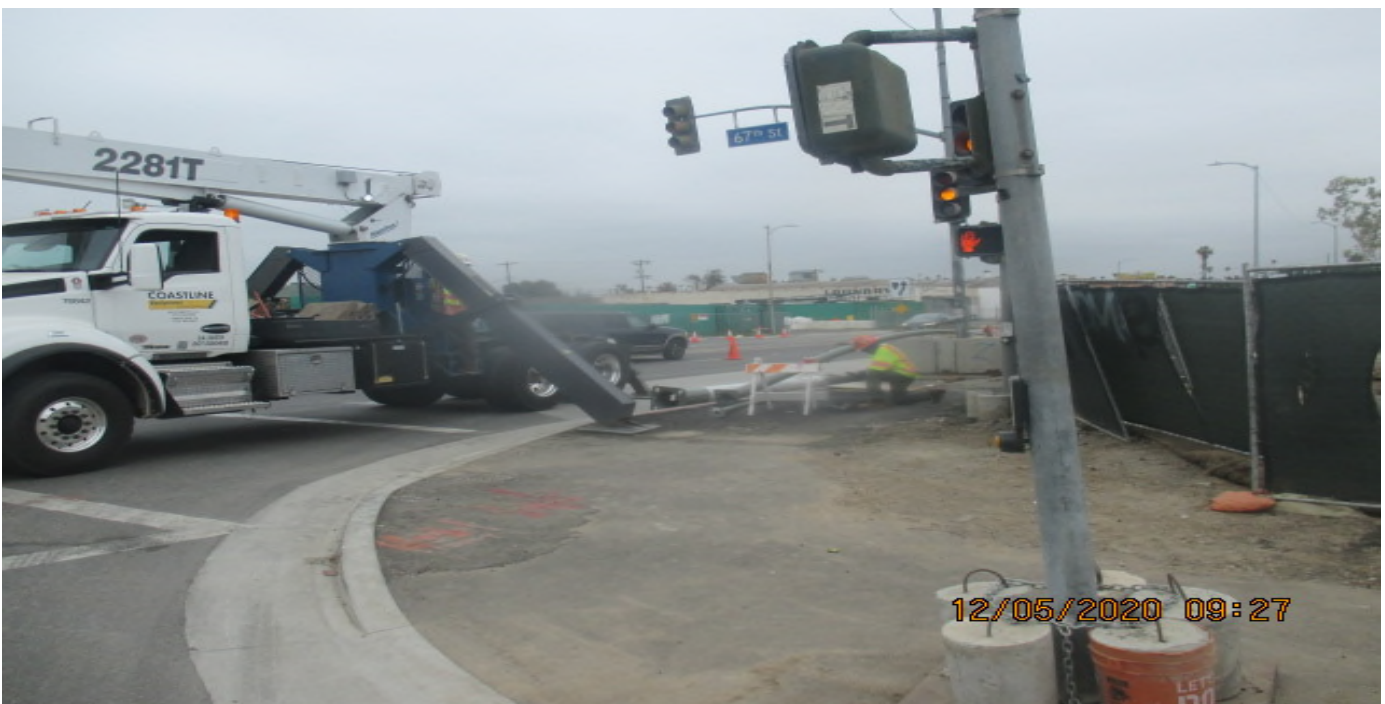
UG3 – Installing street light pole on the southwest corner of 67th St and Crenshaw Blvd. 5/12/20
