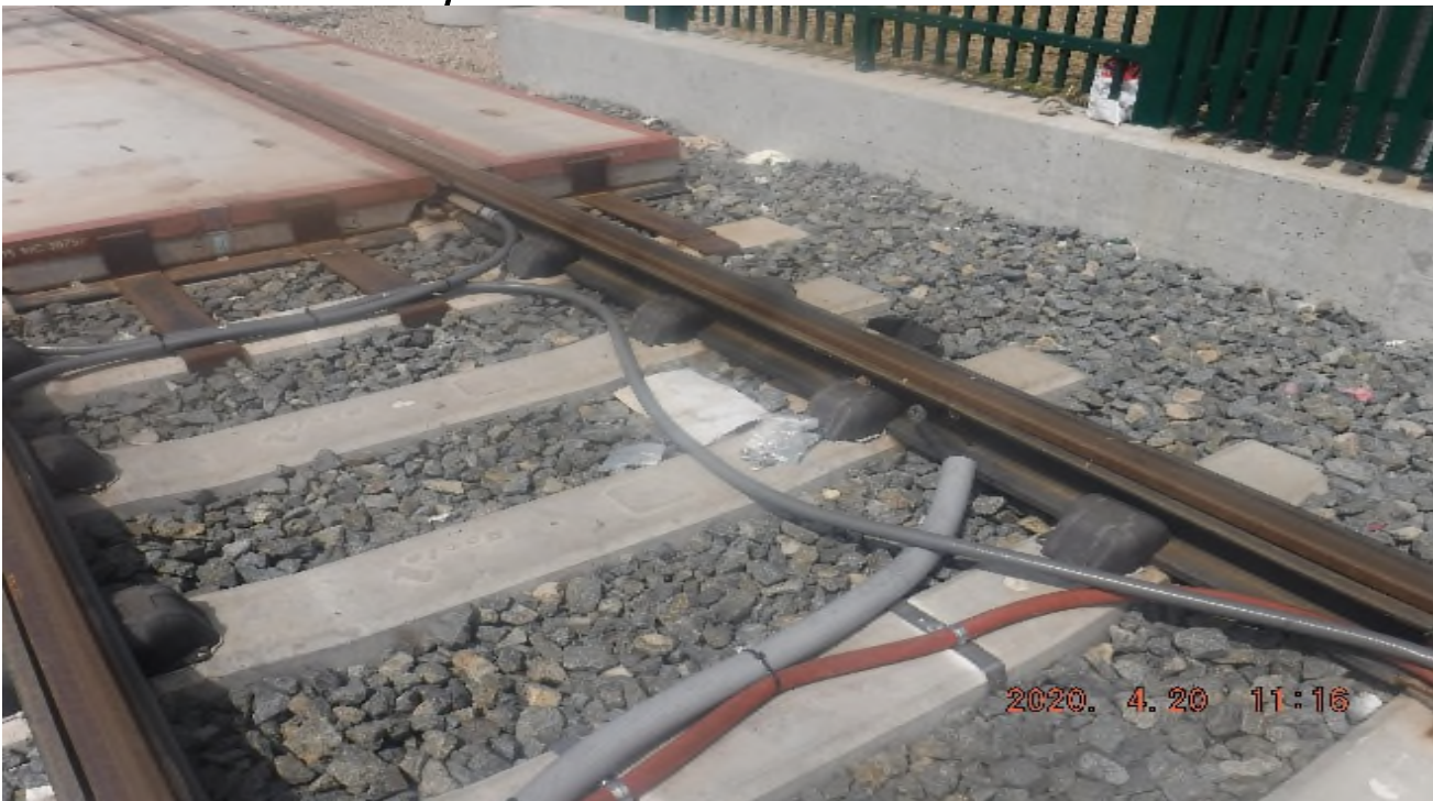
Florence/High St. - STA 257+25 TK#3/SB looking south – system work north end High St at grade Xing.
