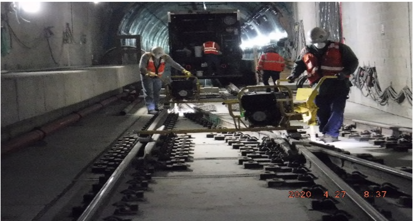
UG-4- STA 441+80 TK#4/NB looking south – torque DF fasteners 8W1LHXO – UG4 Exposition Station.
