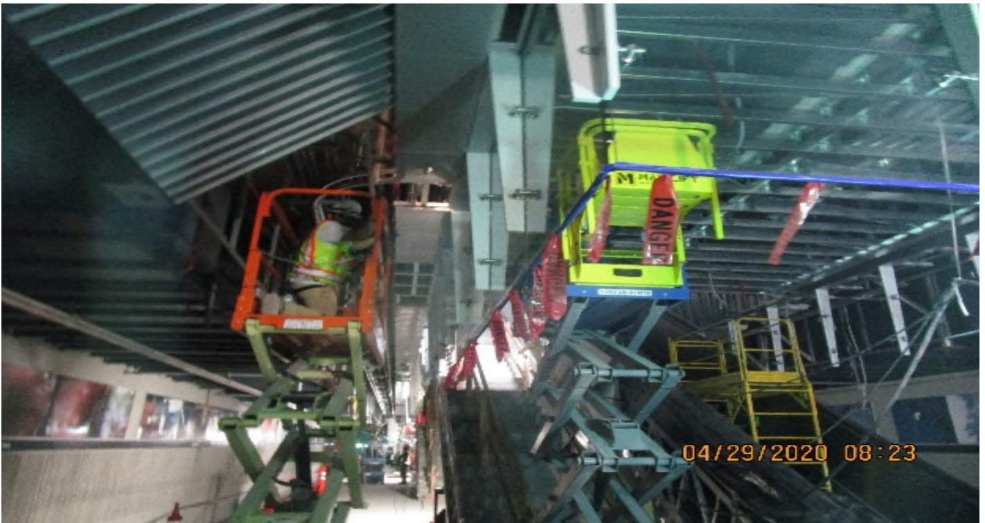
Crenshaw/MLK - MLK, North platform, Northbound continued rough in (3) 2" GRC Radiax cable support conduit, supports & racks.
