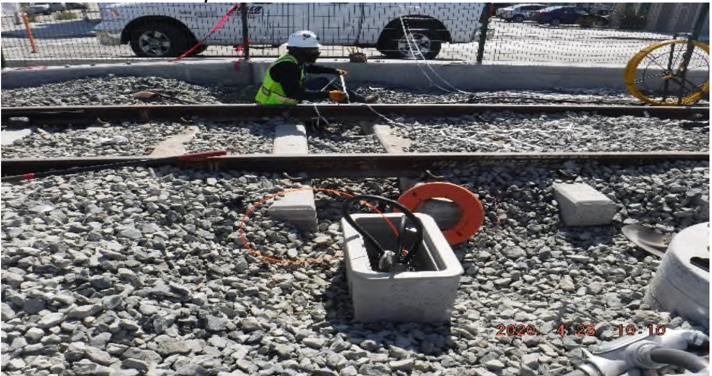
57 th Street - STA 329+90 TK#4/NB looking east – system work with track structure disturbance south of 57th St – PUNCH LIST.
