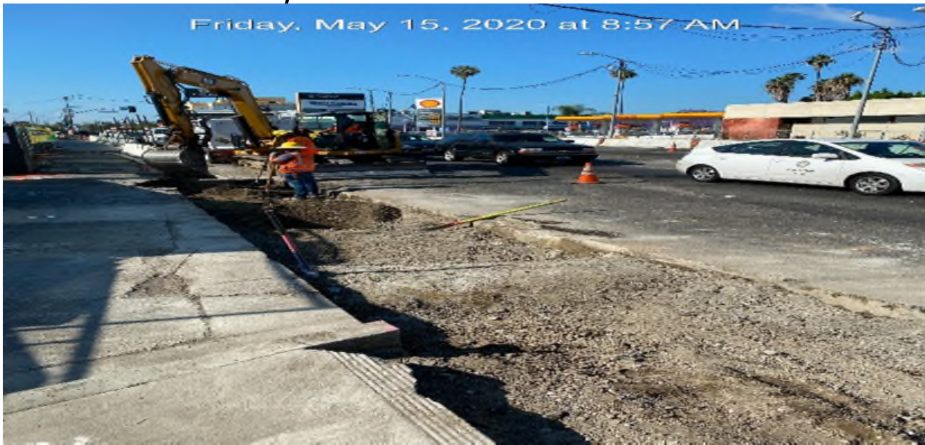
EXPO STATION – Excavating sidewalk for new curb/gutter installation on northbound Crenshaw Blvd between Obama Blvd and Exposition Blvd.
