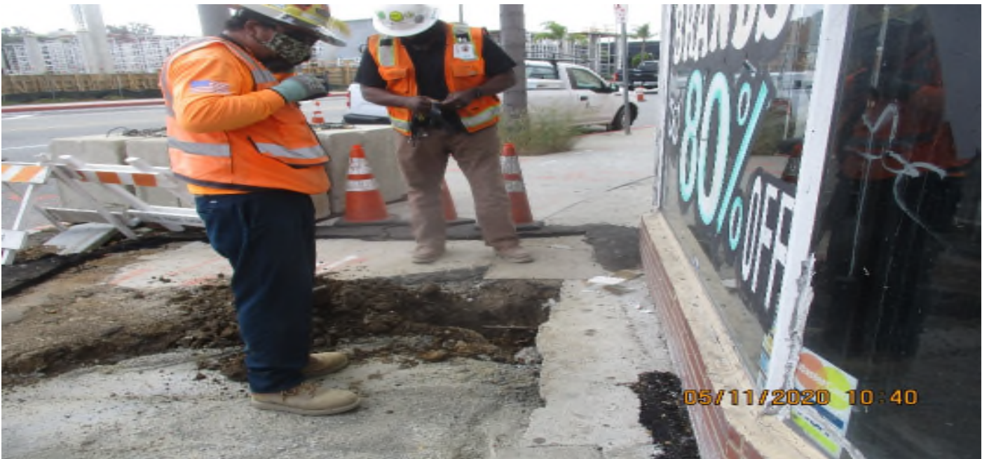
Florence/Brea - WSCC/ Pan Pacific to cut and remove gas line at La Brea and Florence.
