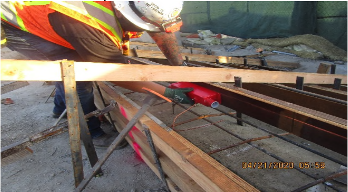
LEIMERT PARK STATION – Began layout of recessed lighting fixtures for planter stair risers on the northwest section of the plaza level.
