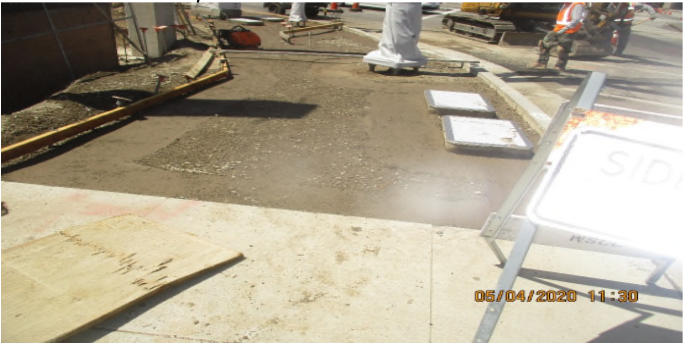
Florence/Brea - WSSC placed SWK concrete at N/W corner of La Brea and Florence.
