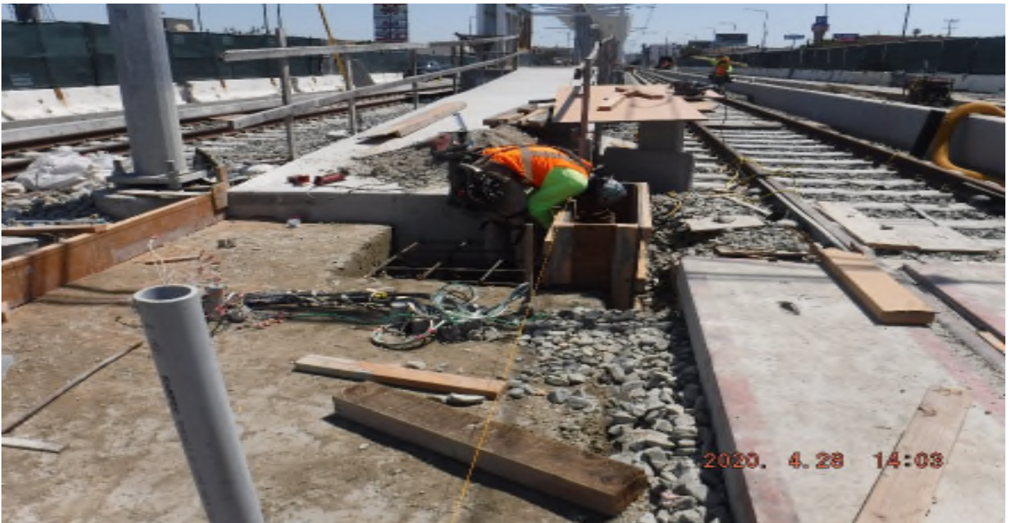
Crenshaw / Slauson - STA 323+00 TK#3/SB looking south – set form and rebar at north end of Slauson Station for future pedestrian pad
