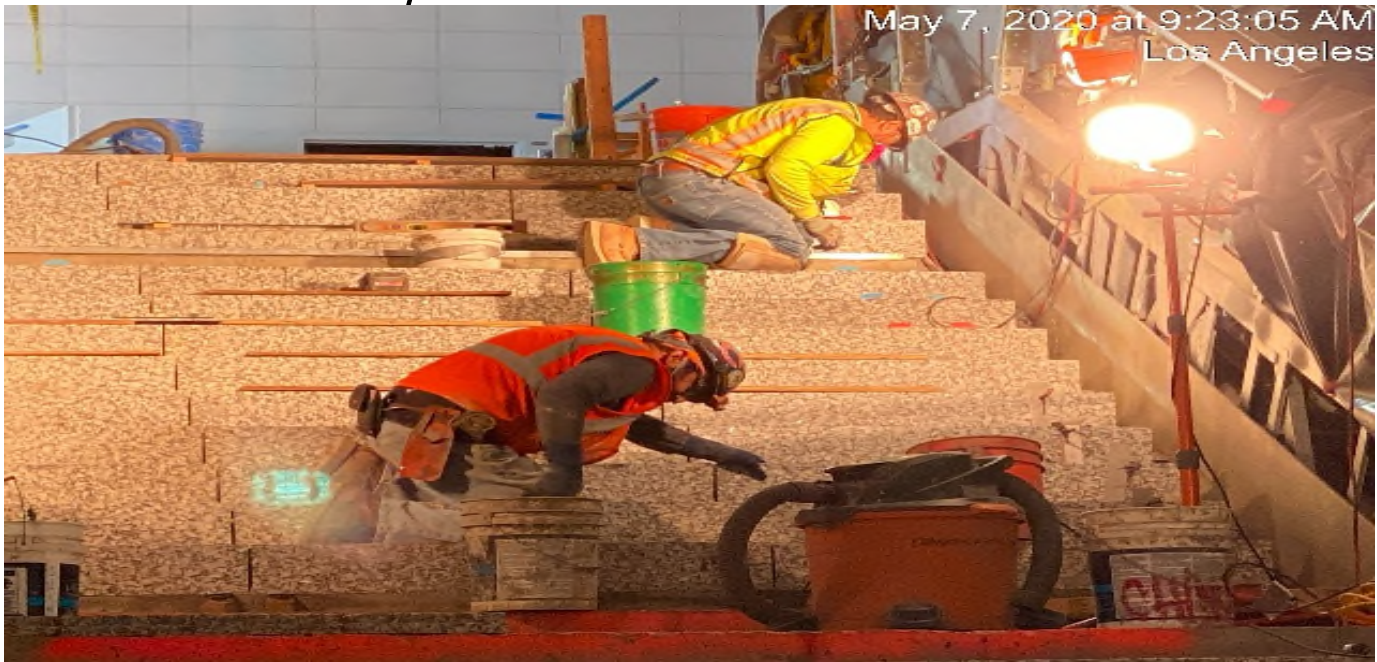
LEIMERT PARK STATION – Continue granite thread and riser installation at the intermediate stair case landing.
