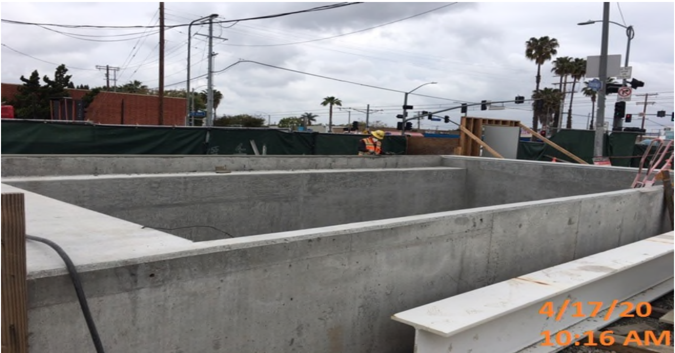
EXPO STATION – Continue surfacing walls of the north emergency ventilation shaft at the plaza level.
