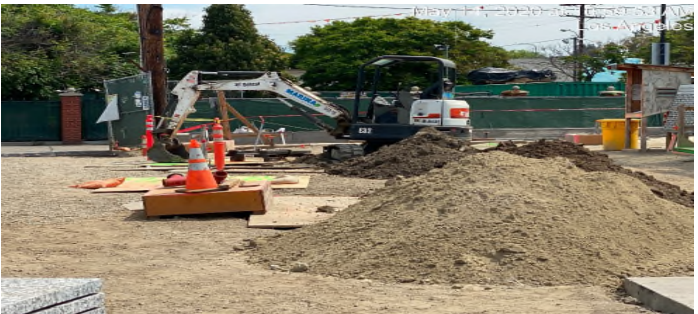
LEIMERT PARK STATION – Continue excavating for palm tree installation at the plaza.
