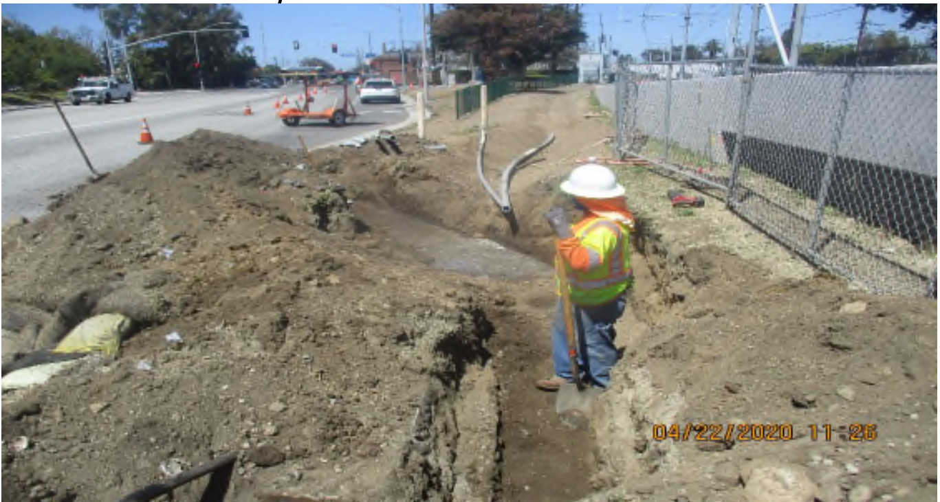
Florence/High St. - Select Electric Place TS conduit at E/B Florence and High St.
