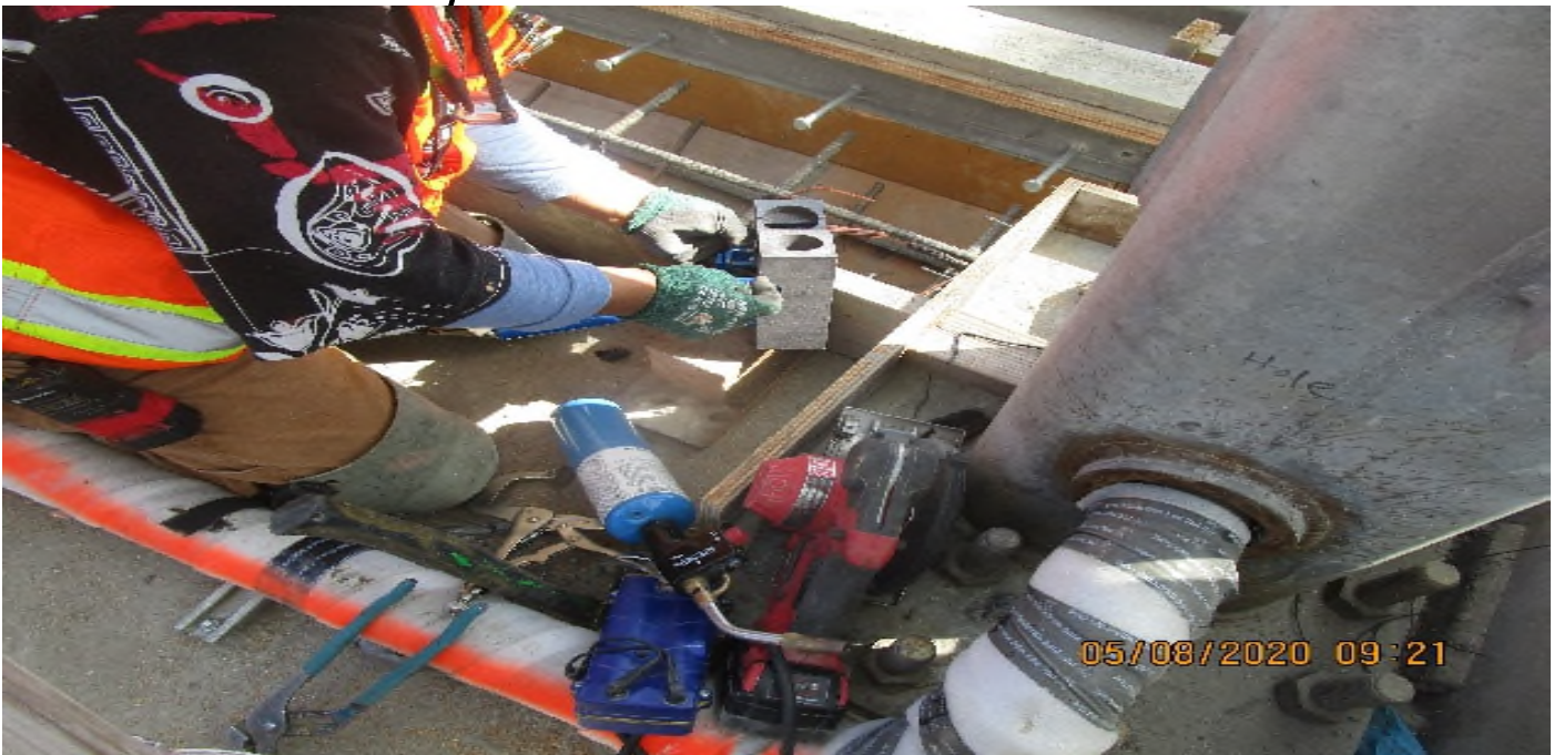
LEIMERT PARK STATION – Embedding whips to the north emergency exit hatch doors at the plaza level.
