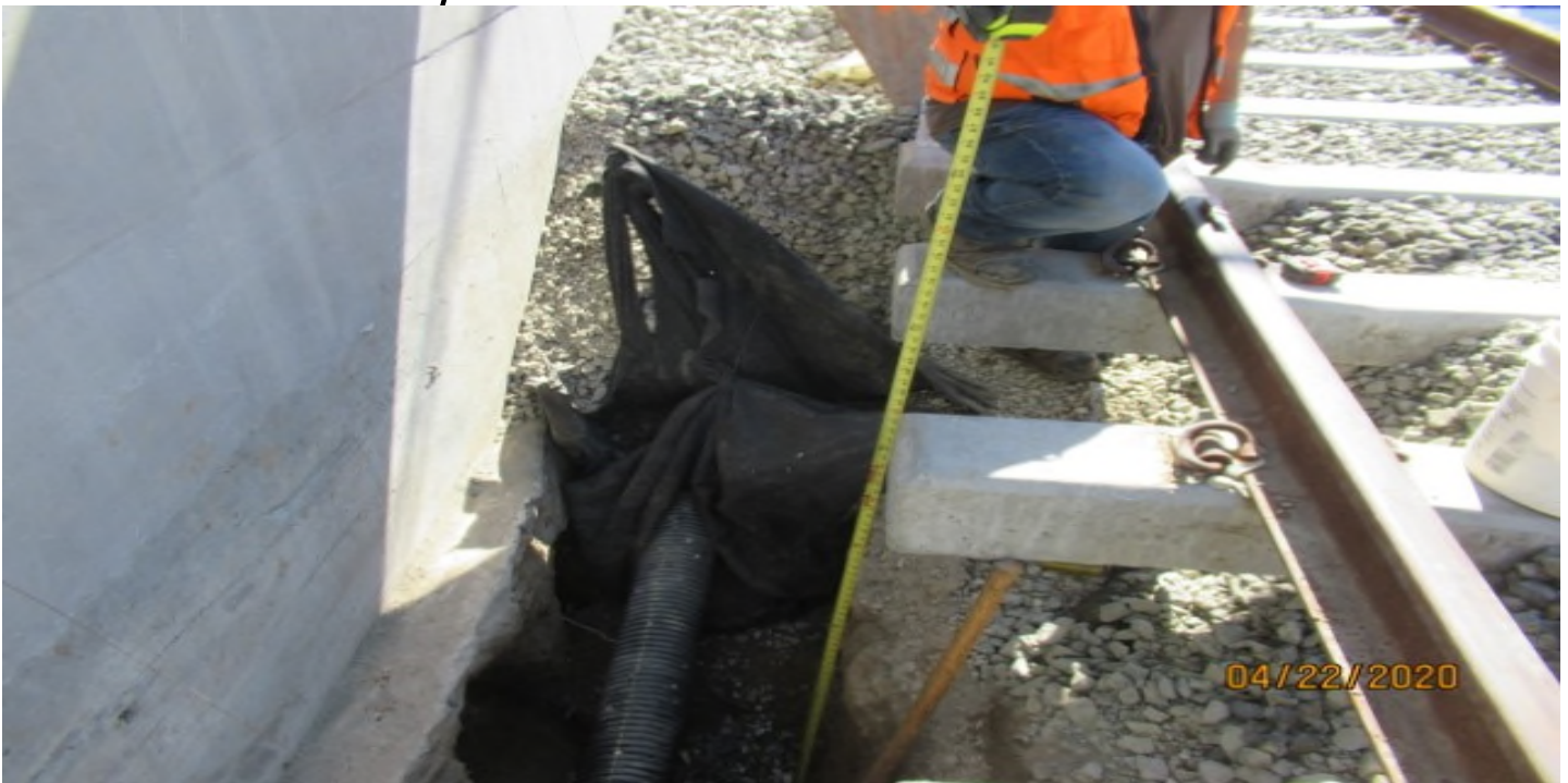
AVIATION/CENTURY- Mesurment of 66+inches from bottom of excavation hole to top of tie on SB #3 track STA 178+00 Segment B1 (looking north) Rework,This will need to be re-tamped – century
