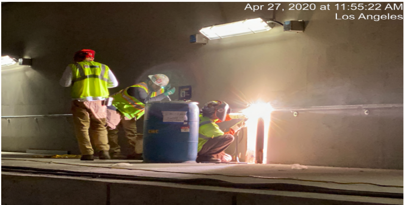
UG4 – Continue handrail installation for the emergency walkways along the northbound tunnel at Sta 378+00.
