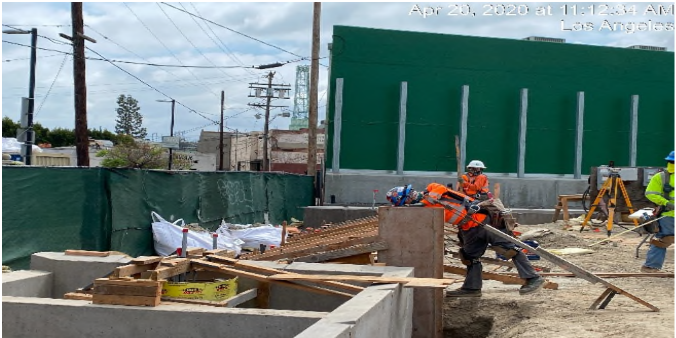
LEIMERT PARK STATION – Continue formwork for the planter stair risers on the northwest section of the plaza level.
