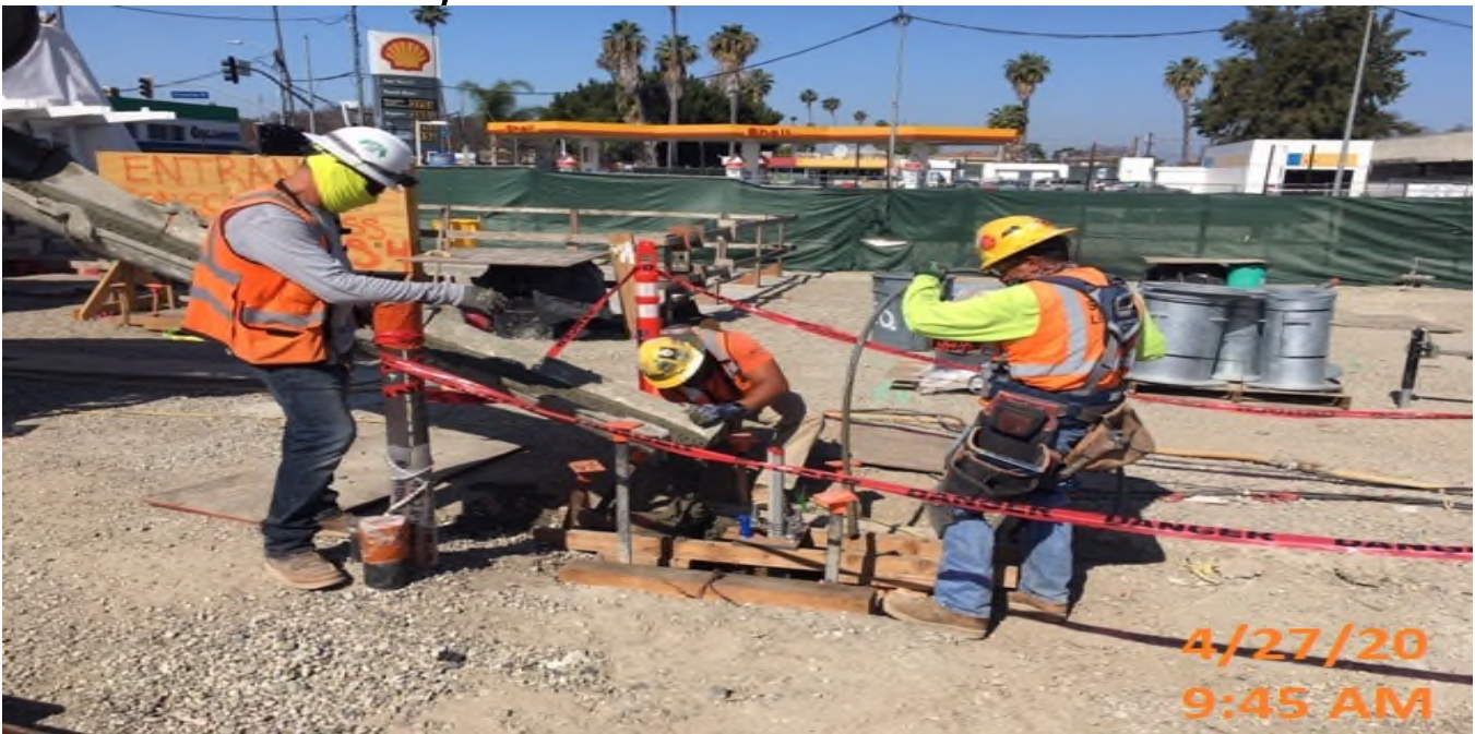
EXPO STATION – Placing concrete for the light pole foundations at the plaza level.
