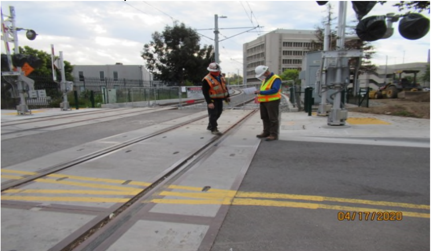
Florence/Ivy – WSCC & Metro inspector's gathering data for rail gouges at Ivy Ave grade crossing STA 189+00 (looking north)
