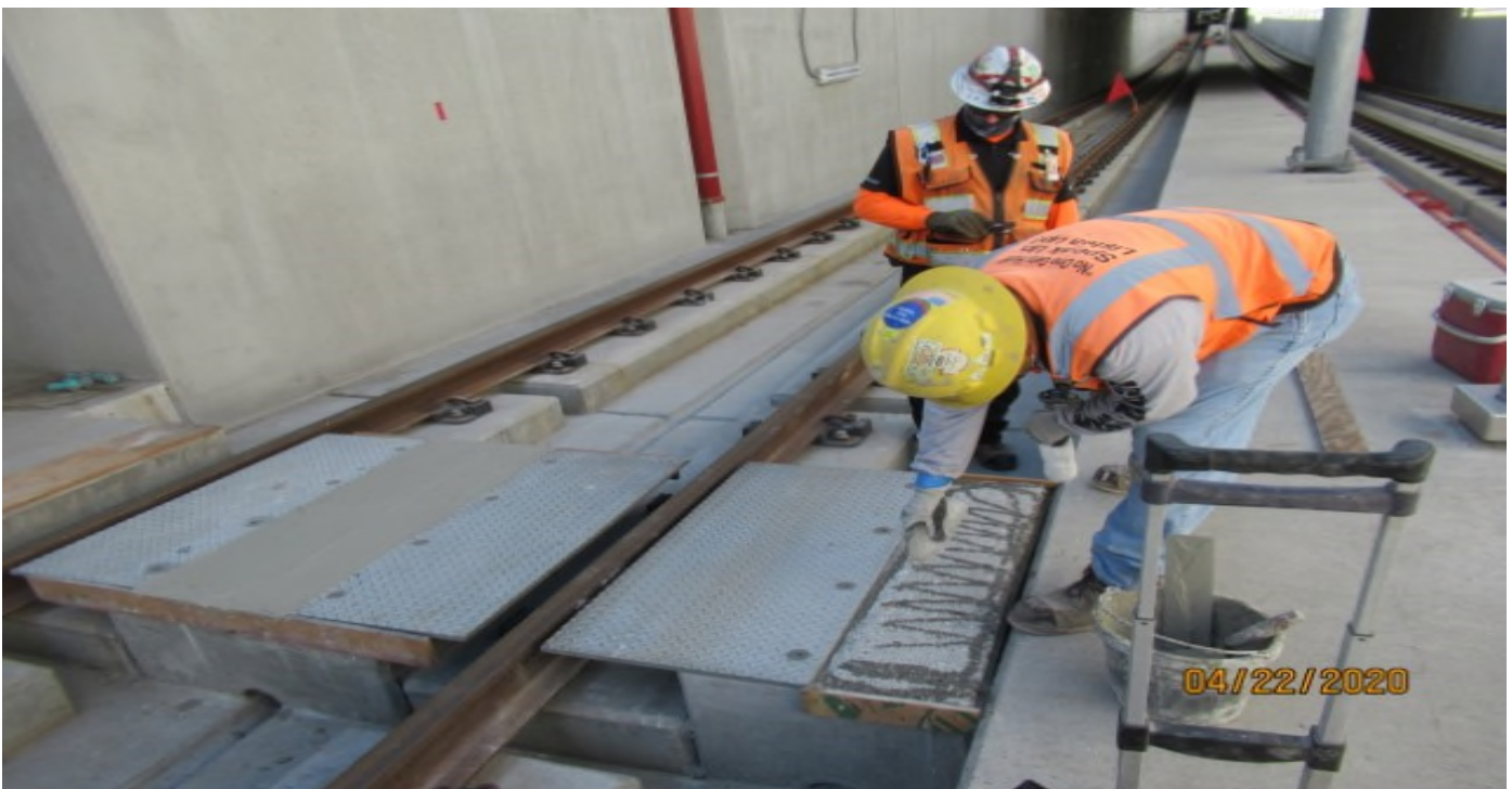
UG1 - WSCC concrete foreman leveling foundation for plates on emergency walkway in UG1 NB #4 track STA 56+50 (looking south) Rework
