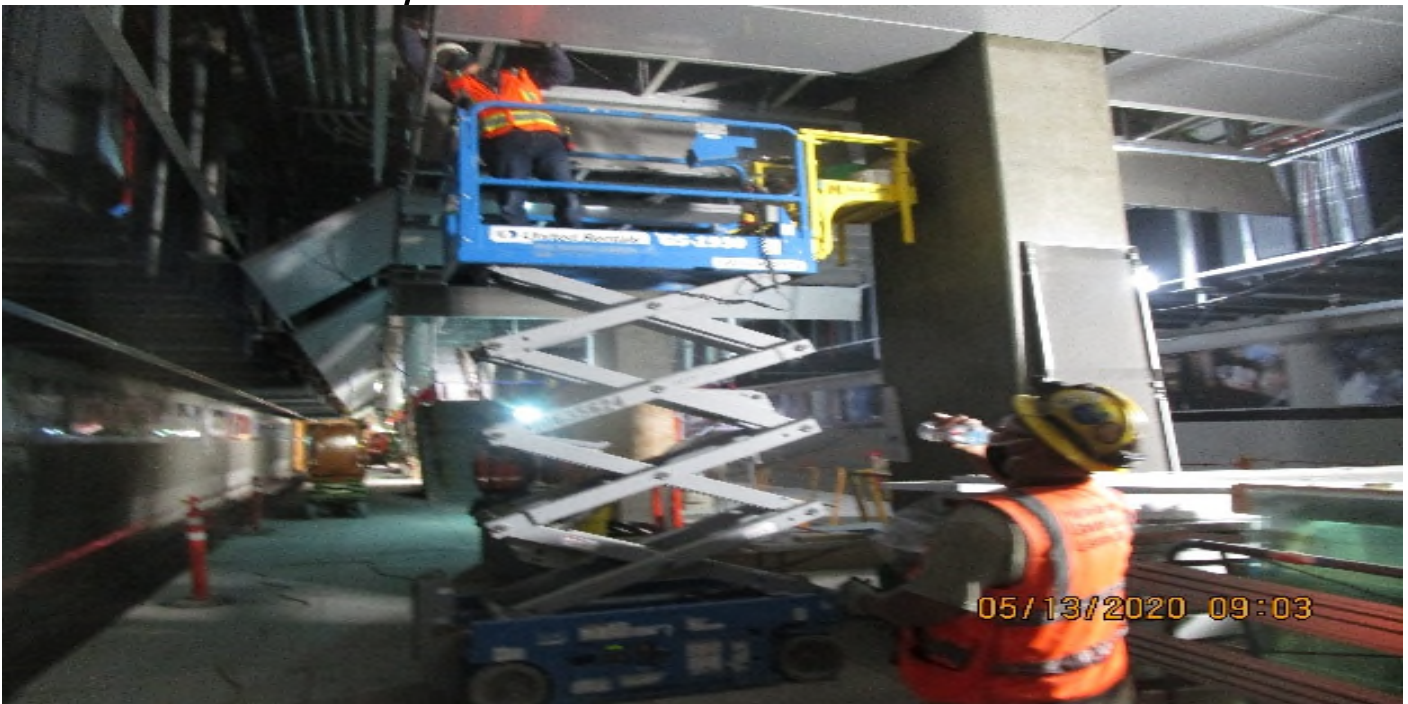
LEIMERT PARK STATION – Began installing ceiling light fixtures at the platform level.
