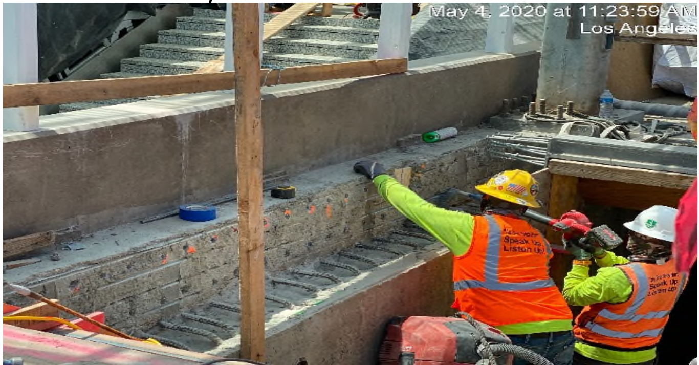
LEIMERT PARK STATION – Drilling and doweling for the north emergency exit hatch doors at the plaza level.
