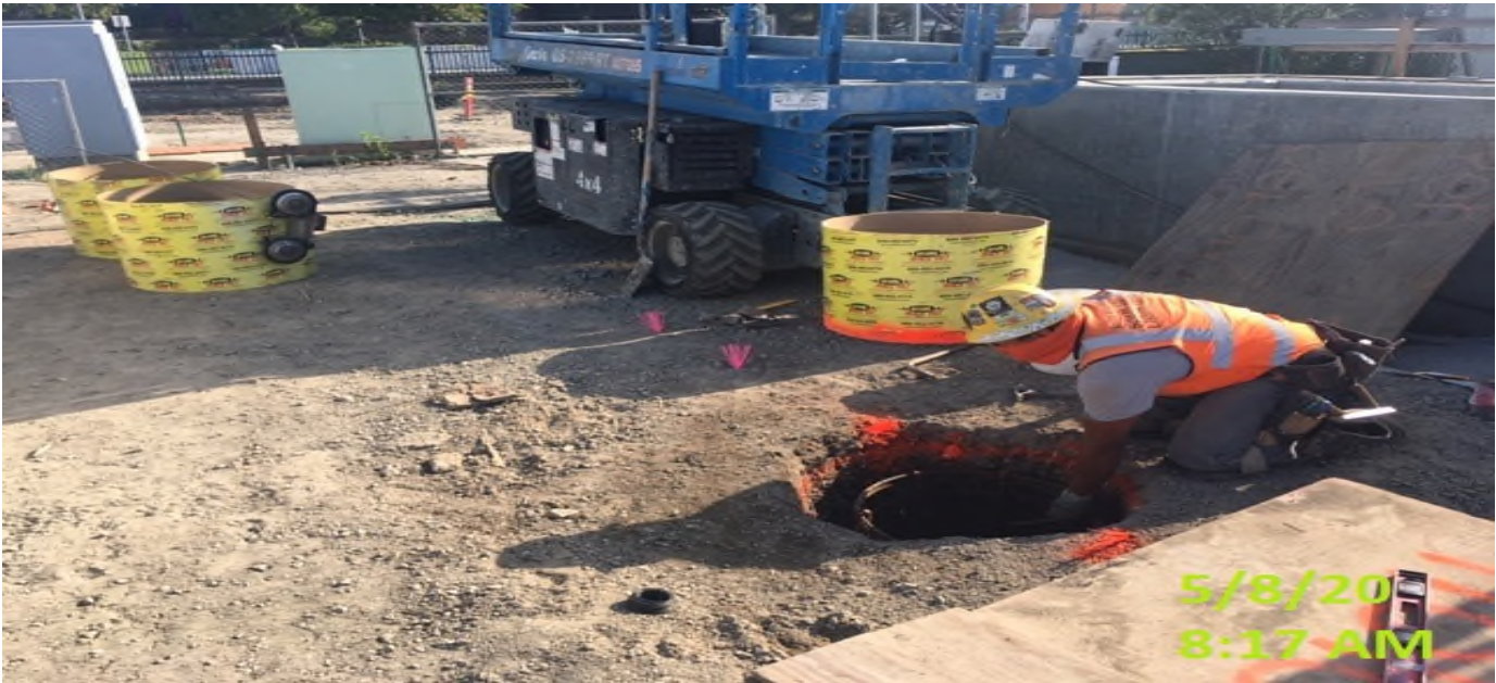
EXPO STATION – Began sonotube formwork for plaza lighting foundations at the plaza level.
