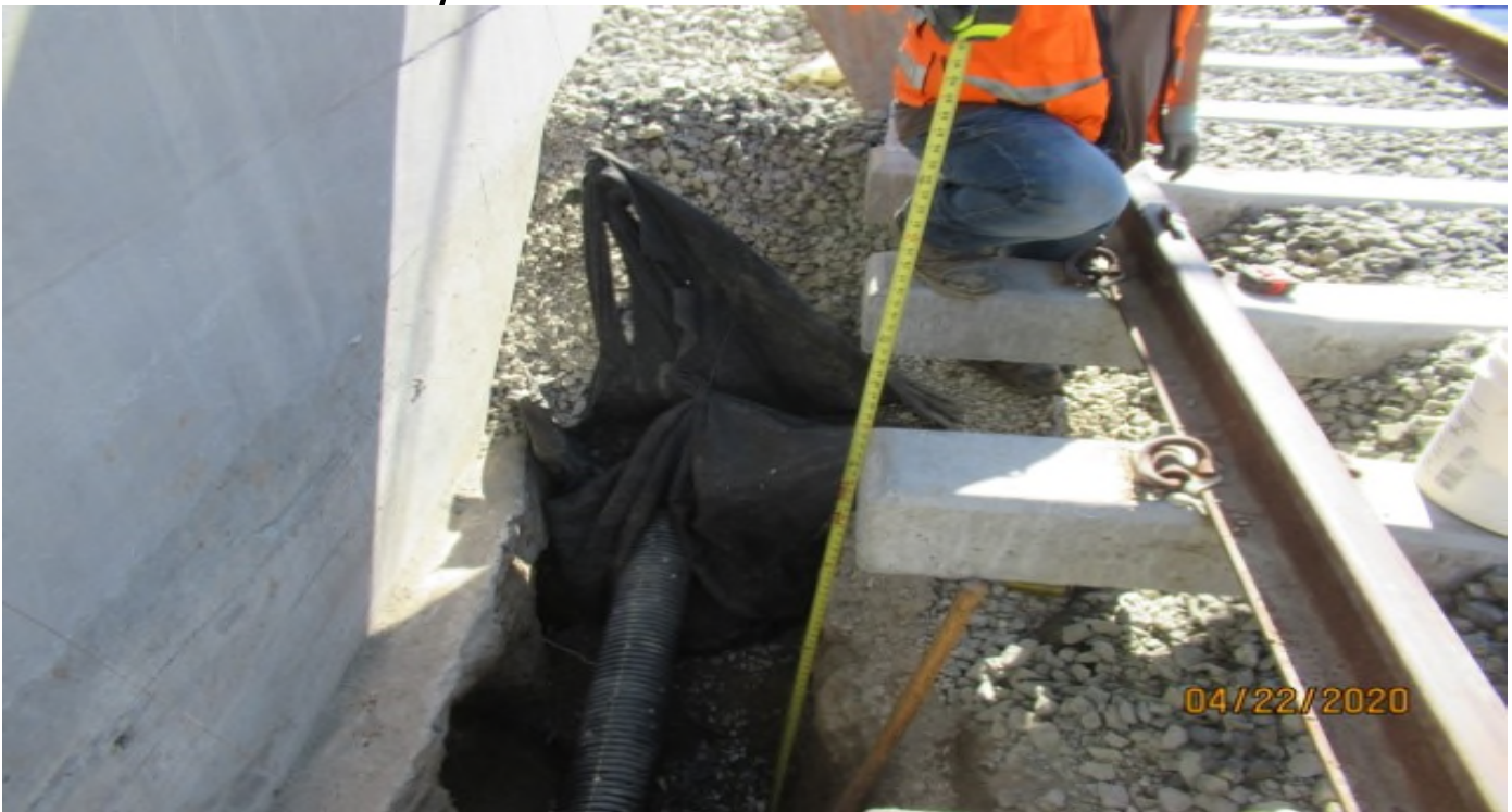
Aviation/Century – Measurement of 66+inches from bottom of excavation hole to top of tie on SB #3 track STA 178+00 Segment B1 (looking north) Rework, This will need to be re-tamped – century
