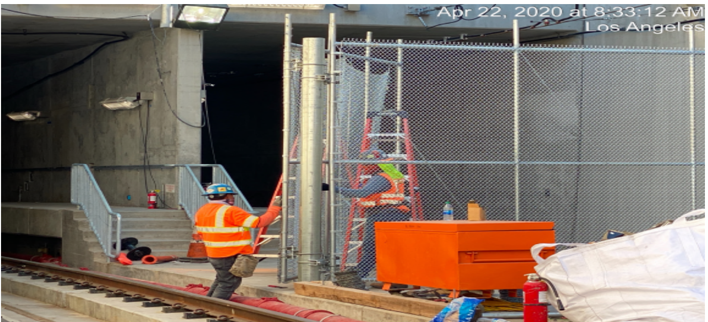
UG3 – Continue installing chain link fencing for both north and southbound tracks at the south end portal entrance.
