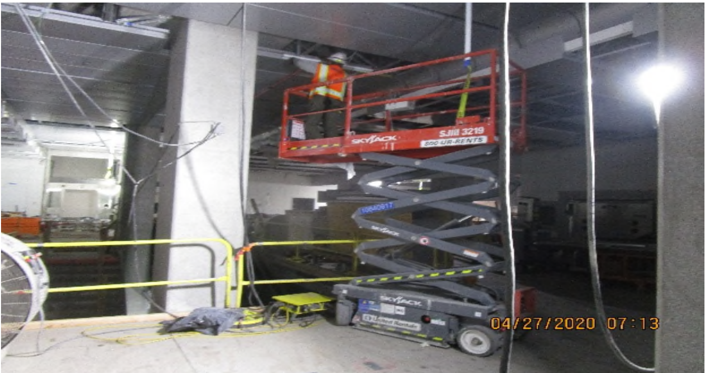
LEIMERT PARK STATION – Continue installing ceiling light fixtures at the concourse level.
