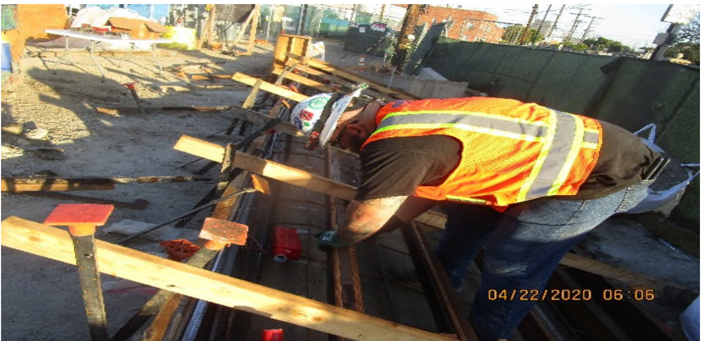
LEIMERT PARK STATION – Continue embedded and ramp lighting fixture installation for planter stair risers on the northwest section of the plaza level.
