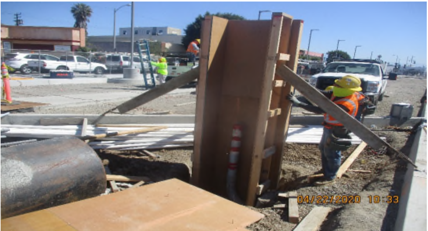
Florence/West – Carpenter Crew Form For emergency generator receptacle pedestal at center of West Station.
