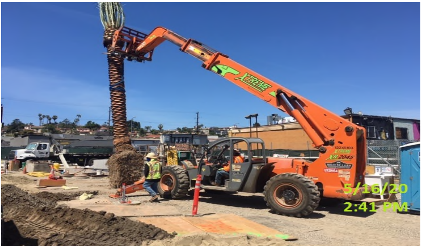
LEIMERT PARK STATION – Continue excavating and began palm tree installation at the plaza.
