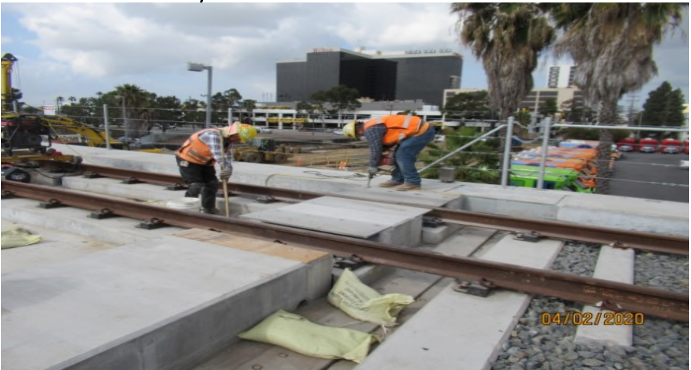
Aviation/Century – WSCC working on emergency walkway foundations Century-Aviation bridge SB #3 track STA 74+60 (looking west) Rework
