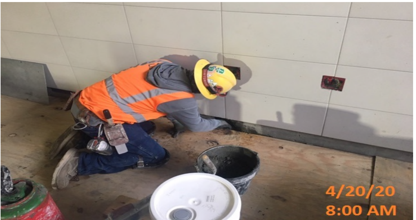
Crenshaw/MLK - MLK – WSCC crew patching voids prior to base cove tile install.
