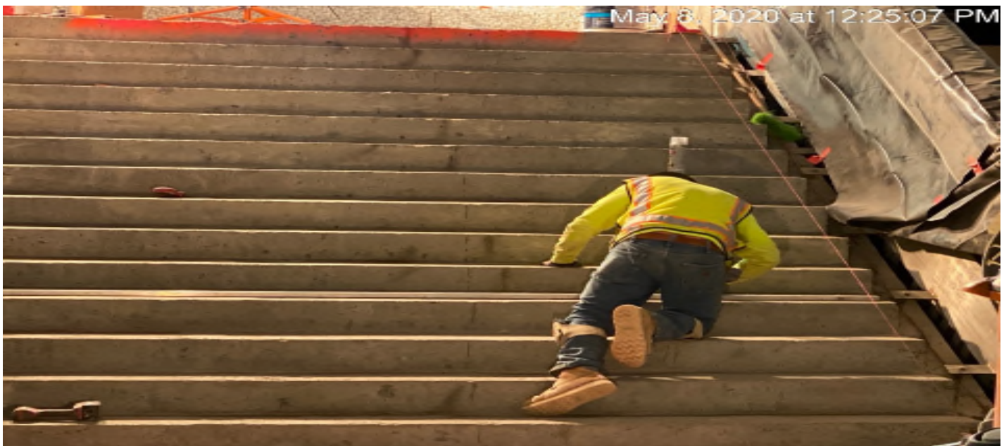
LEIMERT PARK STATION – Continue granite thread and riser installation at the intermediate stair case landing.
