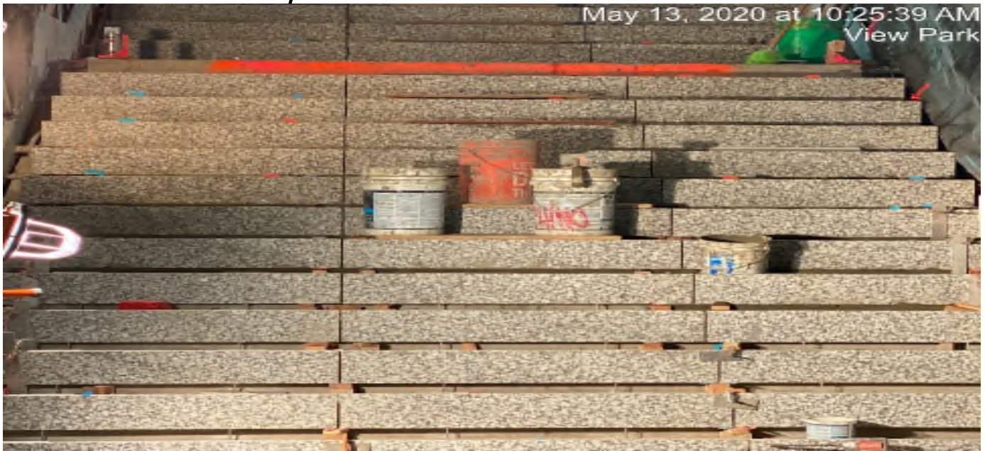
LEIMERT PARK STATION – Continue granite thread and riser installation at the concourse stair case landing.
