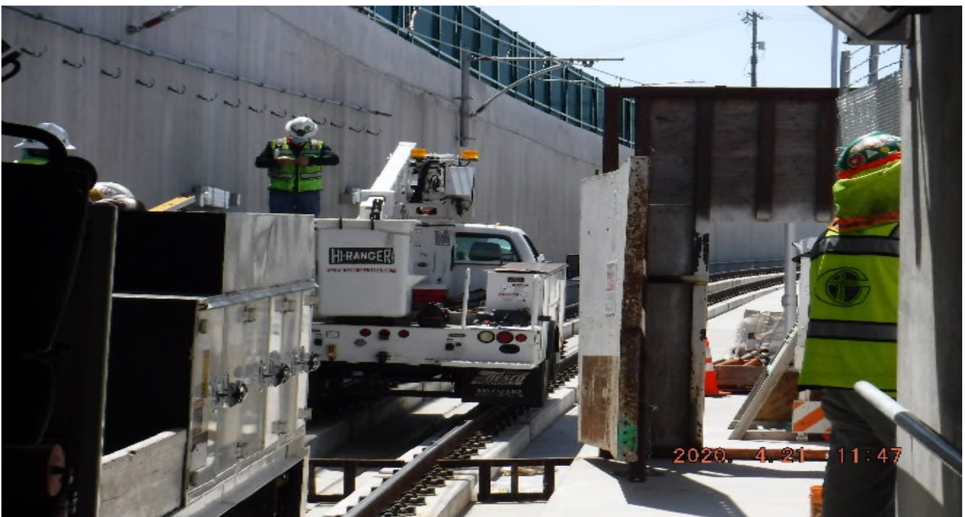
UG-4- STA 371+00 TK#4/NB looking south – OCS work south portal UG4 (48th St).
