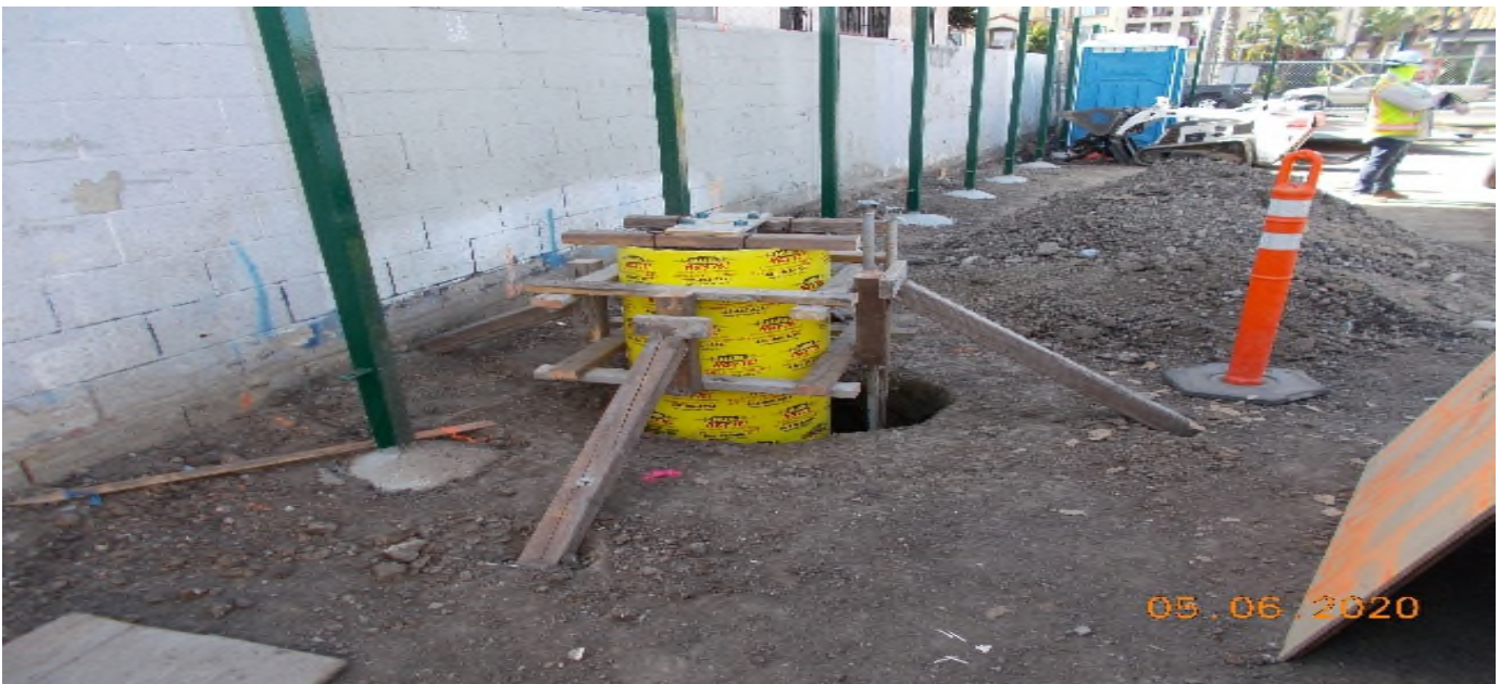
PARK MESA – Continue sonotube formwork and rebar installation for light pole foundations at the northeast corner of TPSS#7 on 60th St & Crenshaw Blvd.
