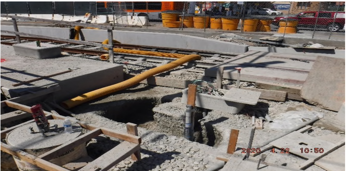
Crenshaw / Slauson - STA 323+00 TK#3/SB looking west – track structure disturbed (between tracks) north end of Slauson Station – PUNCH LIST
