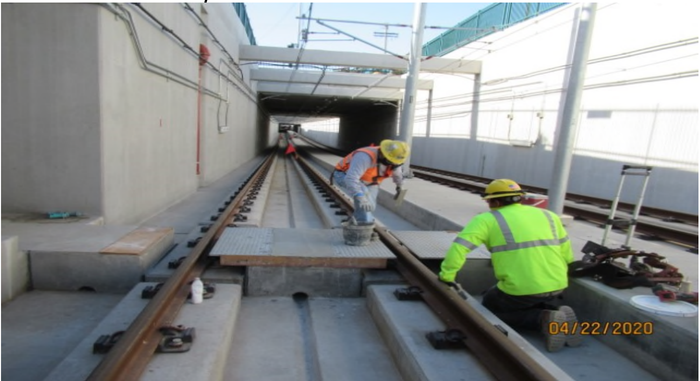
UG1 - WSCC preforming repair work (grouting concrete foundations) on #4 track UG1 STA 56+50 (looking south) Rework.
