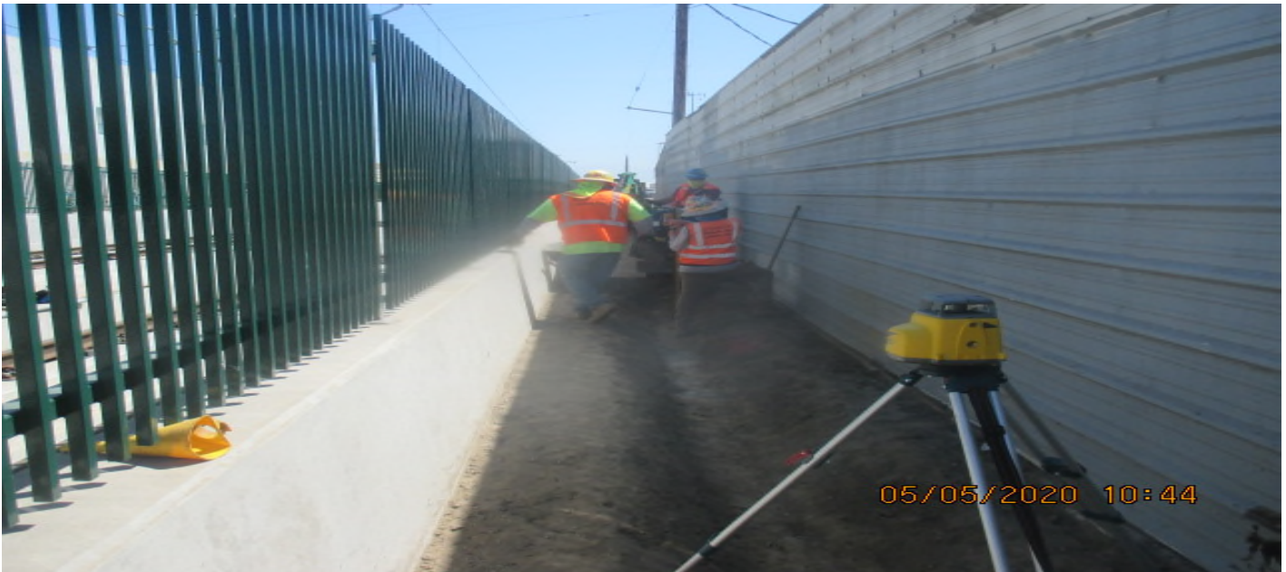
UG3 – Excavating for the culvert drainage system along the northbound barrier wall at Victoria Yard. 5/5/20
