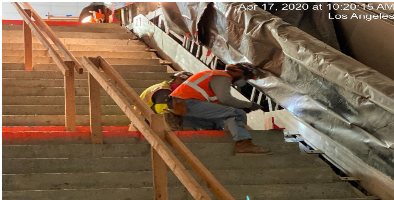
LEIMERT PARK STATION – Continue granite thread and riser installation at the main stair case landing of the plaza level.
