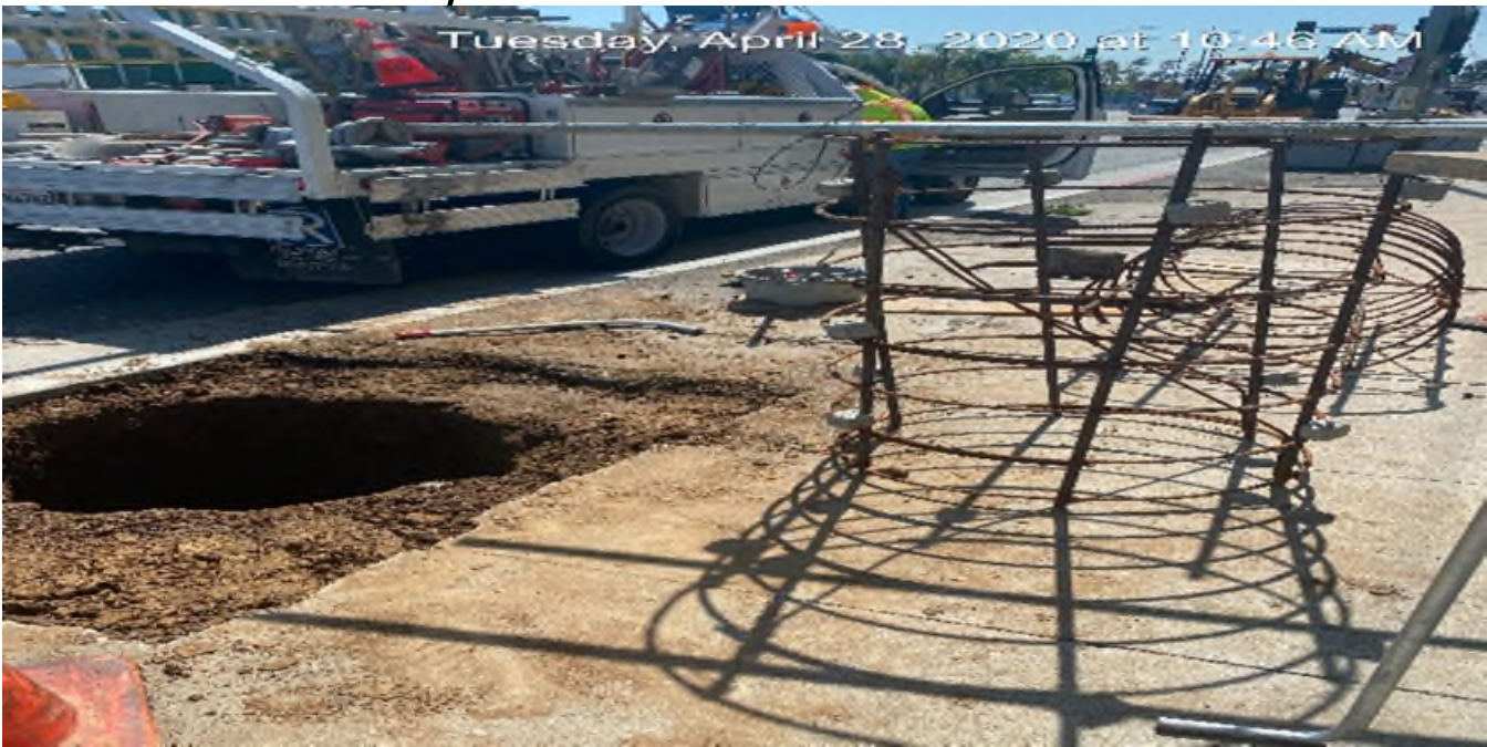
LEIMERT PARK STATION – Began layout for granite installation at the main stair case landing of the plaza level.
