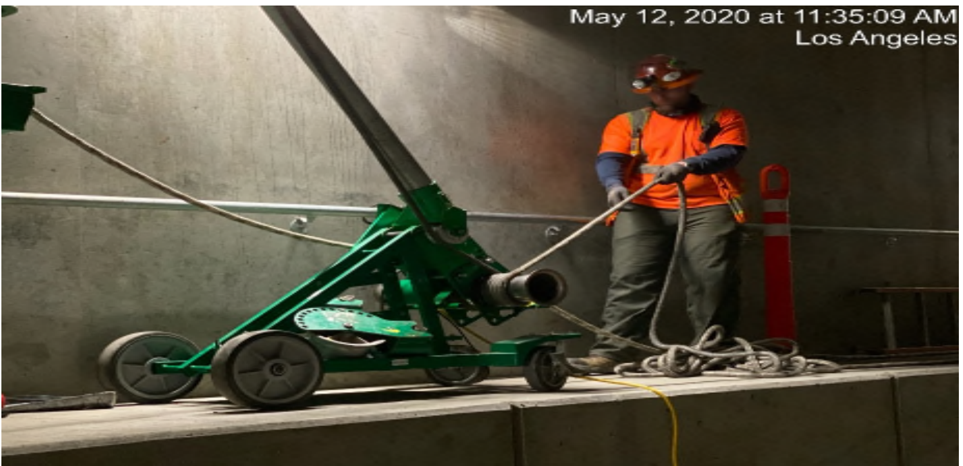
UG3 – Continue pulling permanent power cables for the tunnel booster fans along the northbound tunnel.
