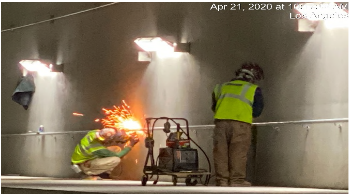
UG4 – Continue handrail installation for the emergency walkways along the southbound tunnel.
