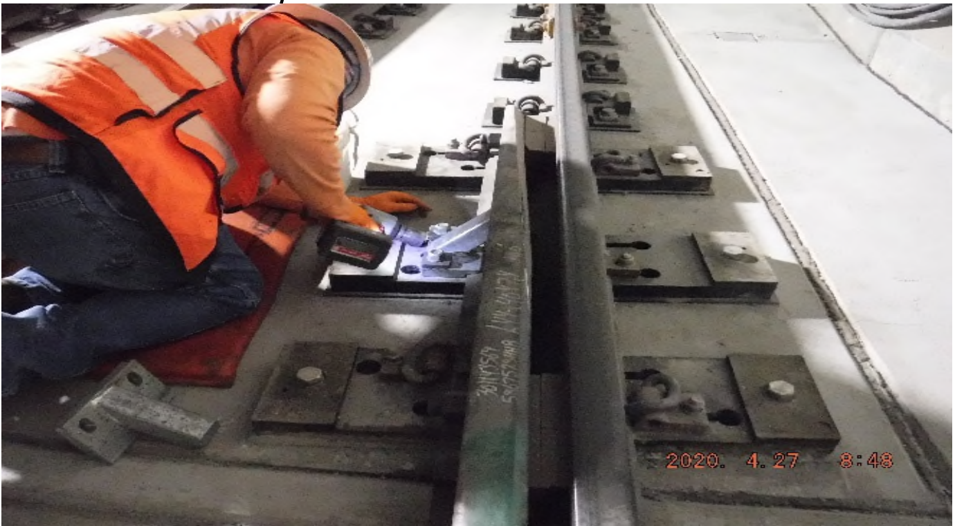
UG-4- STA 440+65 TK#4/NB looking south – set guard rail brackets 8W1LHXO – UG4 Exposition Station
