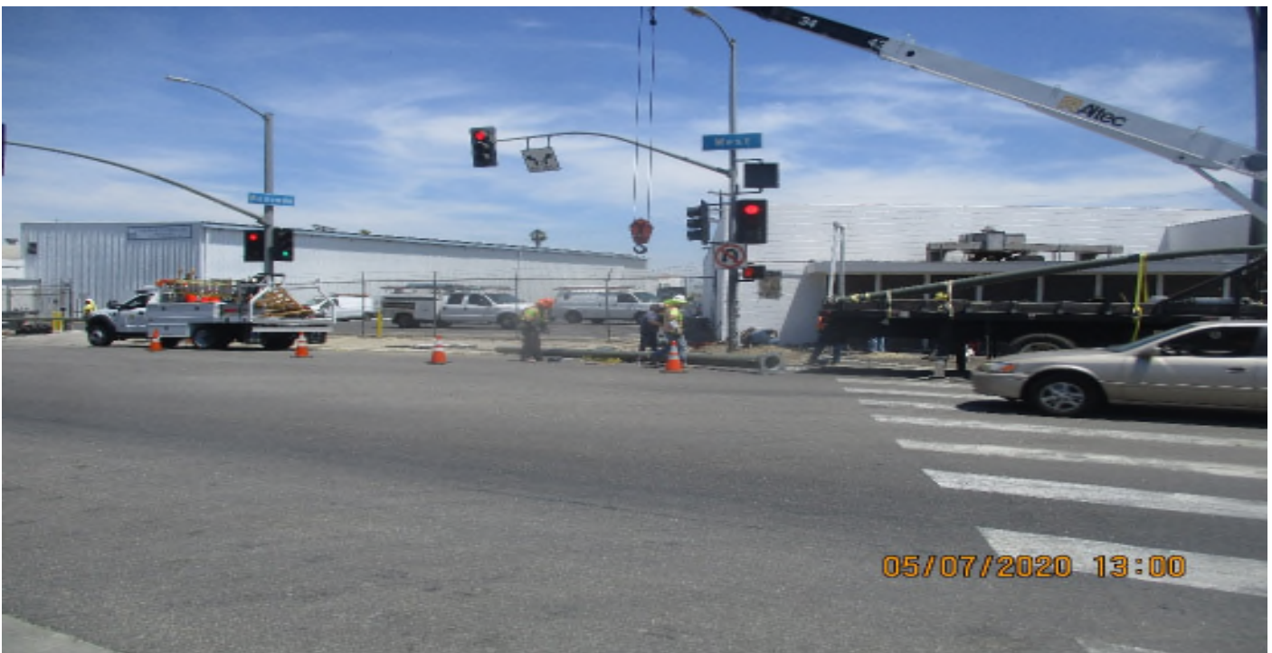
Florence/West – Select Electric Pulling wire and standing poles at Redondo and West St.
