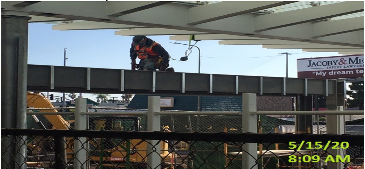
MLK STATION – Installing gutter support for the overhead coiling grille at the main entrance canopy structure.
