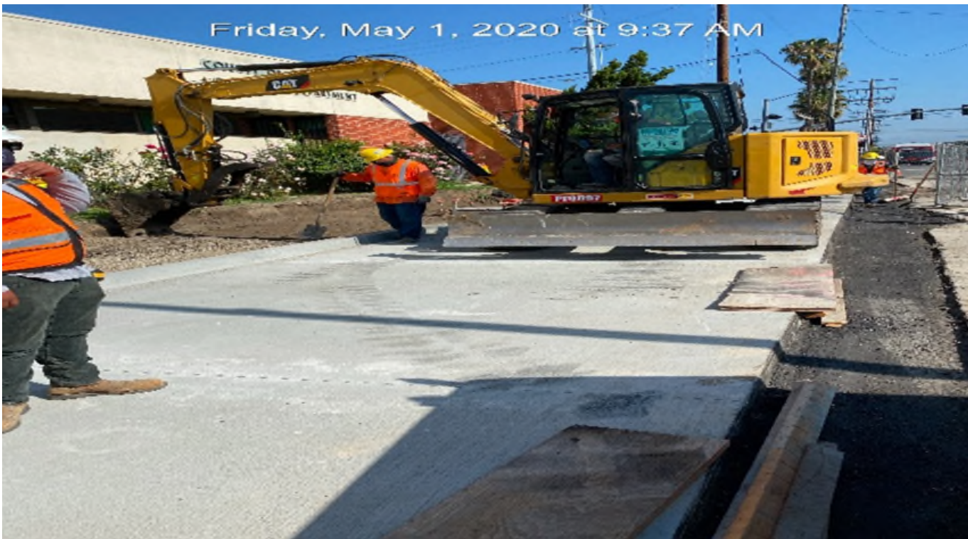
EXPO STATION – Excavating for new sidewalk installation on southbound Crenshaw Blvd between Exposition Blvd and Rodeo Blvd.
