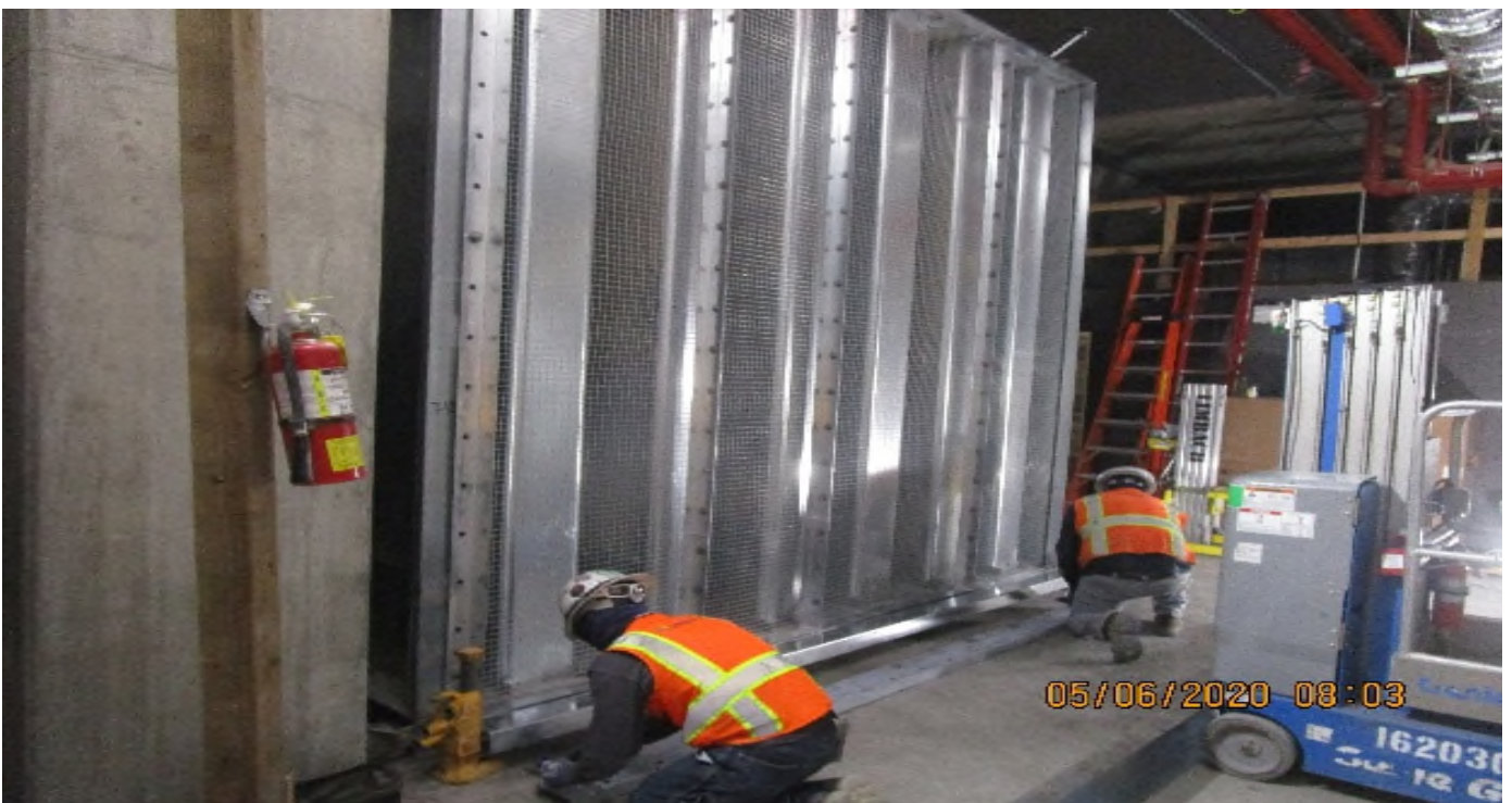
MLK, Emergency fan room (N) C140, continued rough in support hardware TFD-7-122 for (6) damper sections
