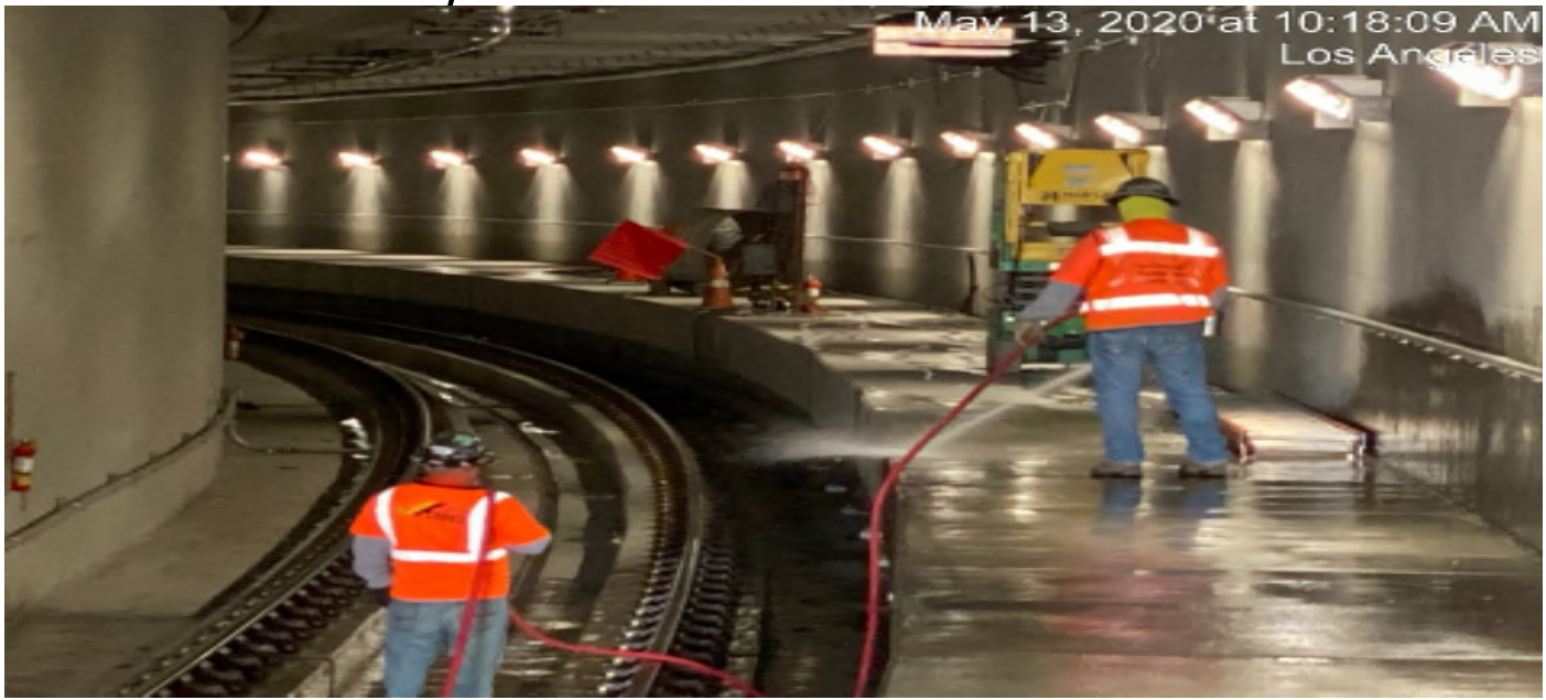
UG4 – Pressure washing concrete between the tracks and cleaning drainage trenches in the southbound tunnel.
