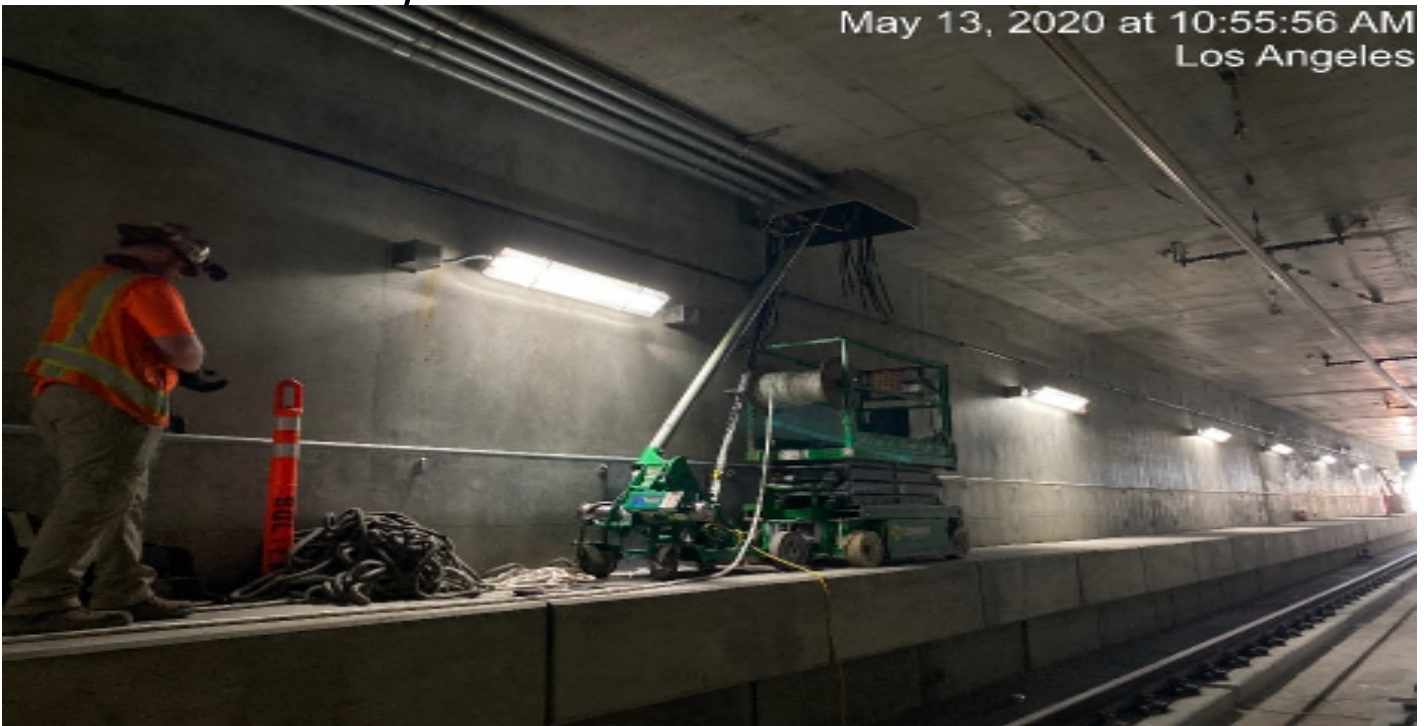
UG3 – Continue pulling permanent power cables for the tunnel booster fans along the northbound tunnel.
