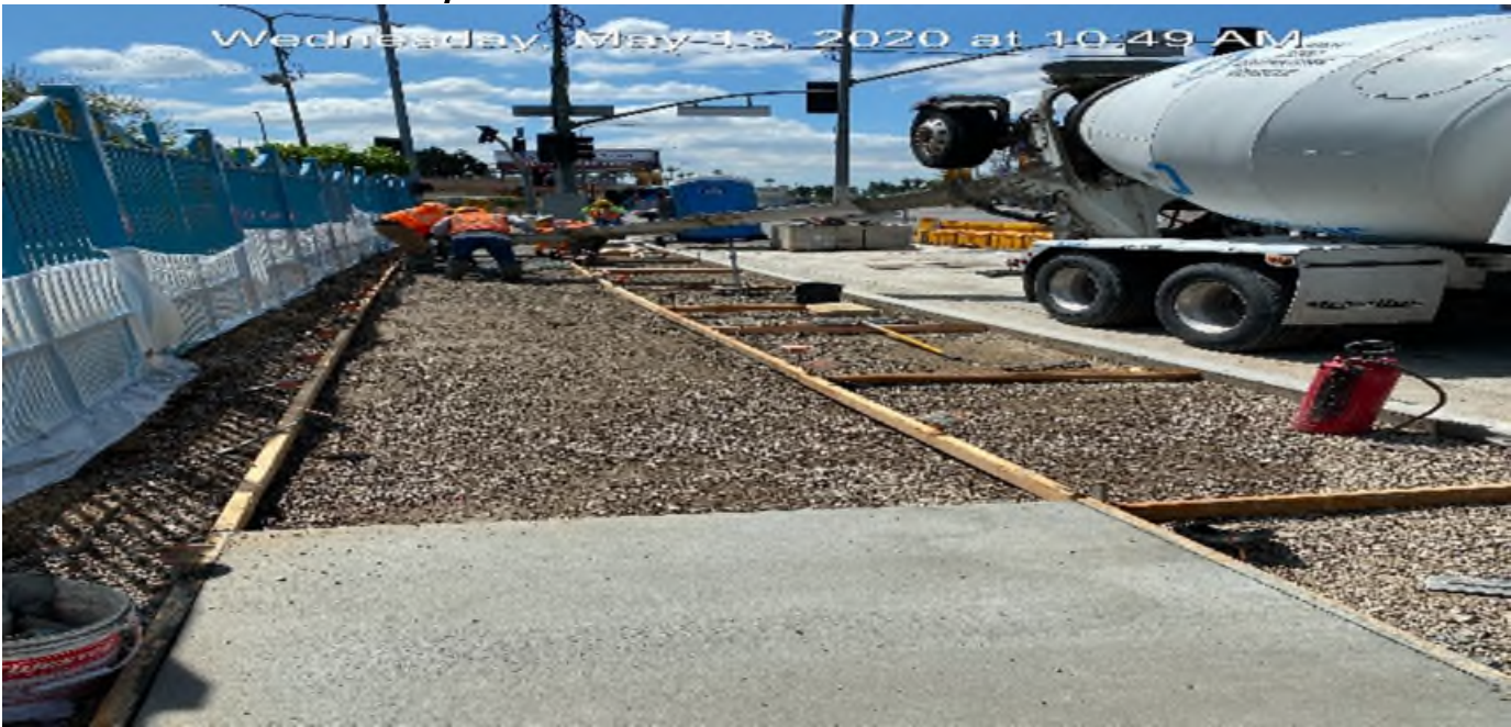
LEIMERT PARK STATION – Built formwork and placed concrete along the northbound sidewalk on Crenshaw Blvd between Vernon Ave and 43rd Pl.
