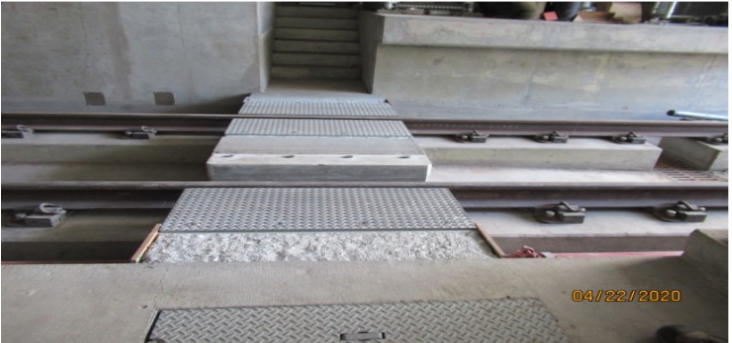
UG1 – UG1 SB #3 track STA 49+78 emergency walkway on-going repair work (looking west) Rework
