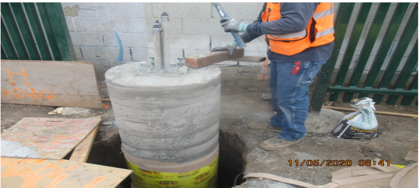
PARK MESA – Stripping forms for the light pole foundations at the northeast corner of TPSS#7 on 60th St & Crenshaw Blvd. 5/11/20
