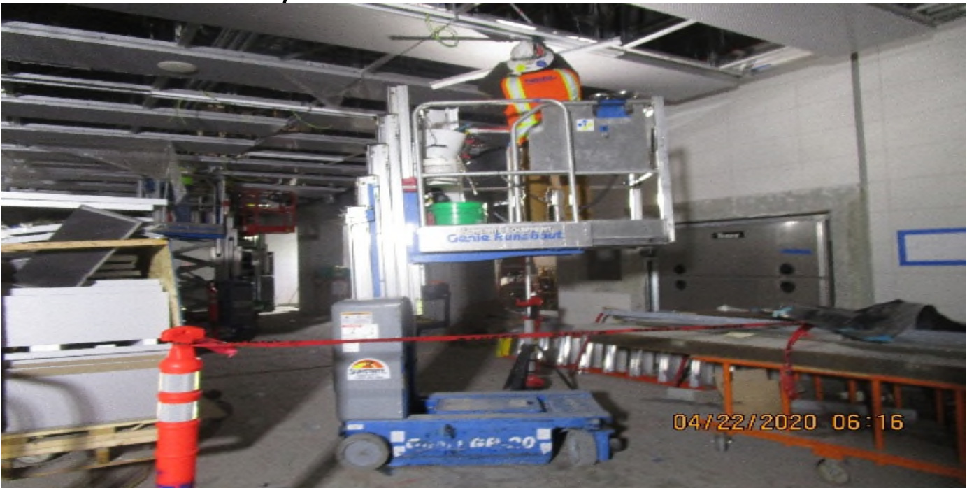
LEIMERT PARK STATION – Continue installing ceiling light fixtures at the concourse level.
