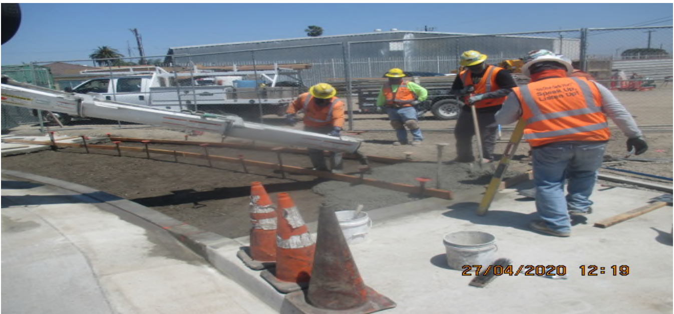
UG3 – Placing concrete for the sidewalk driveway for the Cul-de-sac radius at North Victoria Ave. 4/27/20
