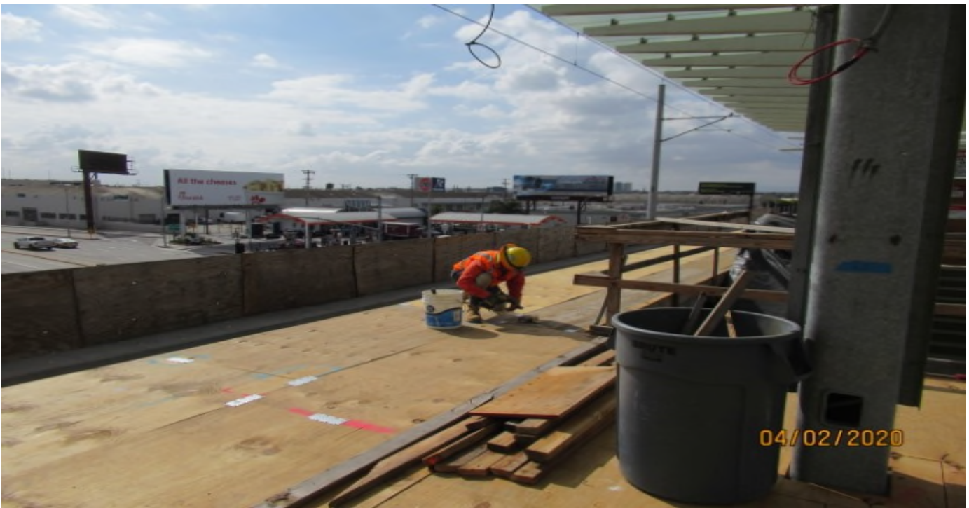
Aviation/Century – WSCC repairing protective plywood on platform at Century-Aviation station (looking southeast)
