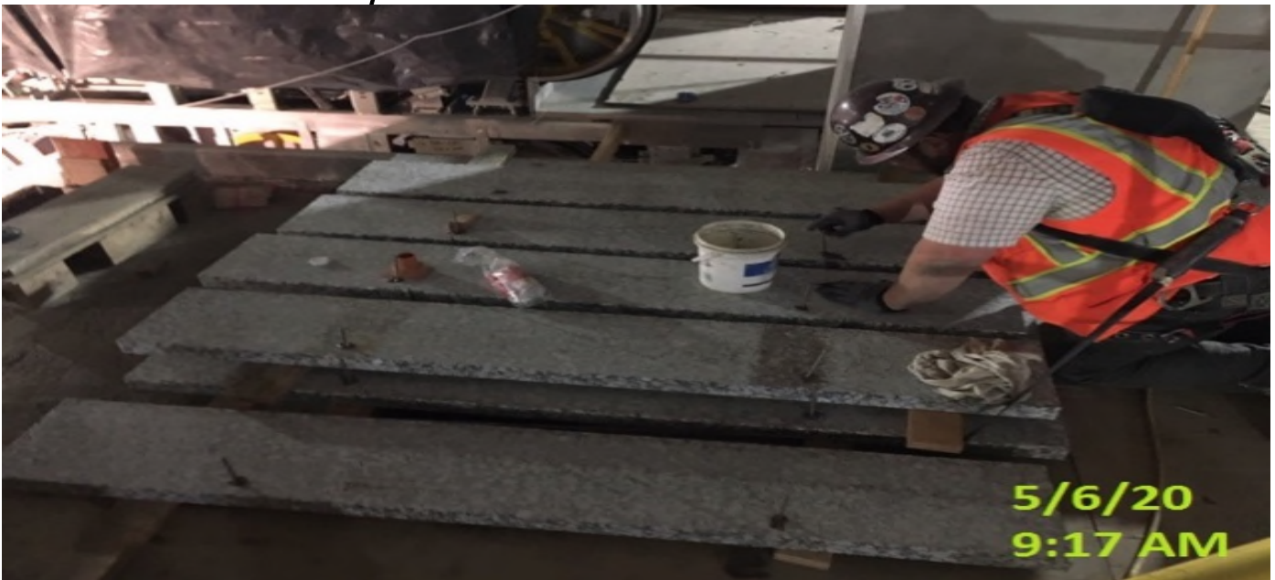
EXPO STATION – Setting dowel pins in granite tread installation for staircase #3 from concourse to platform level.
