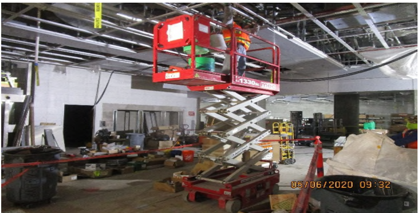
LEIMERT PARK STATION – Continue installing ceiling light fixtures at the concourse level.
