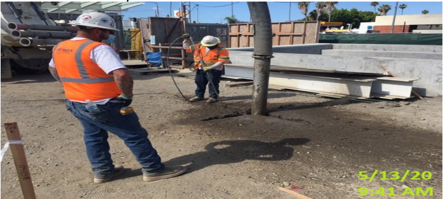
EXPO STATION – Continue potholing for upcoming tree well installation throughout the plaza level.
