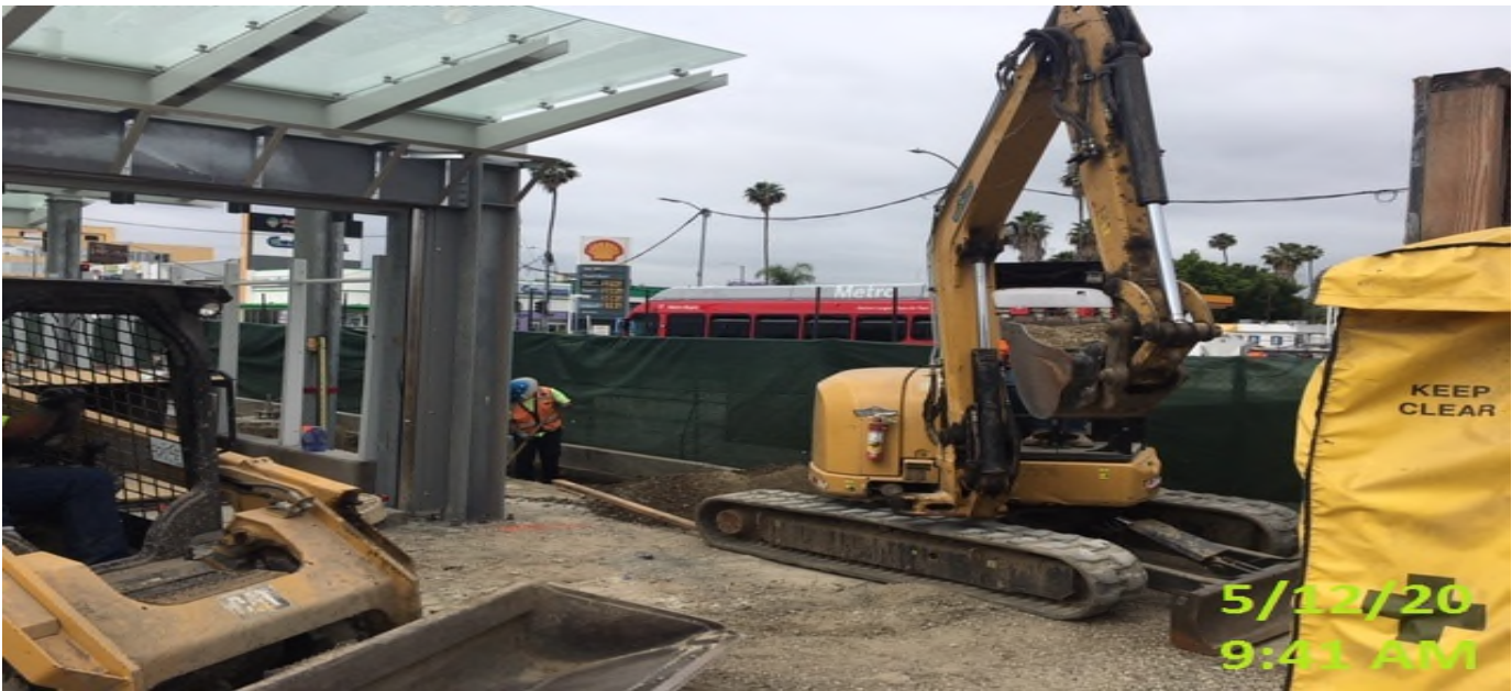
EXPO STATION – Excavating/trenching for upcoming bollard installation on the west side of the plaza level.
