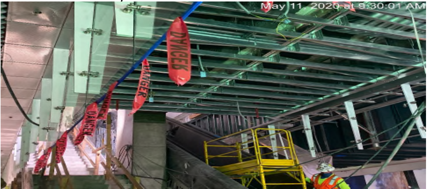
LEIMERT PARK STATION – Began stainless steel cladding installation for the ceiling at the platform level.
