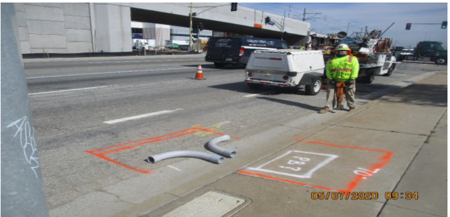
AVIATION/CENTURY - DB Electrical Tie in to existing loop circuits at NB Aviation and 104th St.
