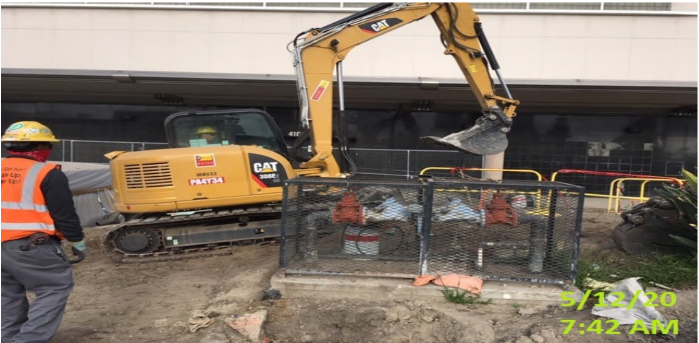
MLK STATION – Continue excavating for 12” HDPE drainage pipe system at the northwest section of the plaza level.
