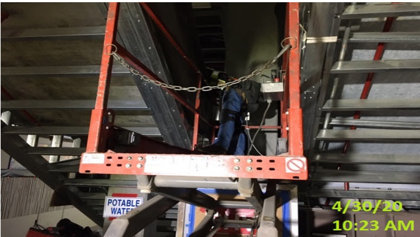
EXPO STATION – Conducting measurements for upcoming layout post installation on staircase #2 at the platform level.
