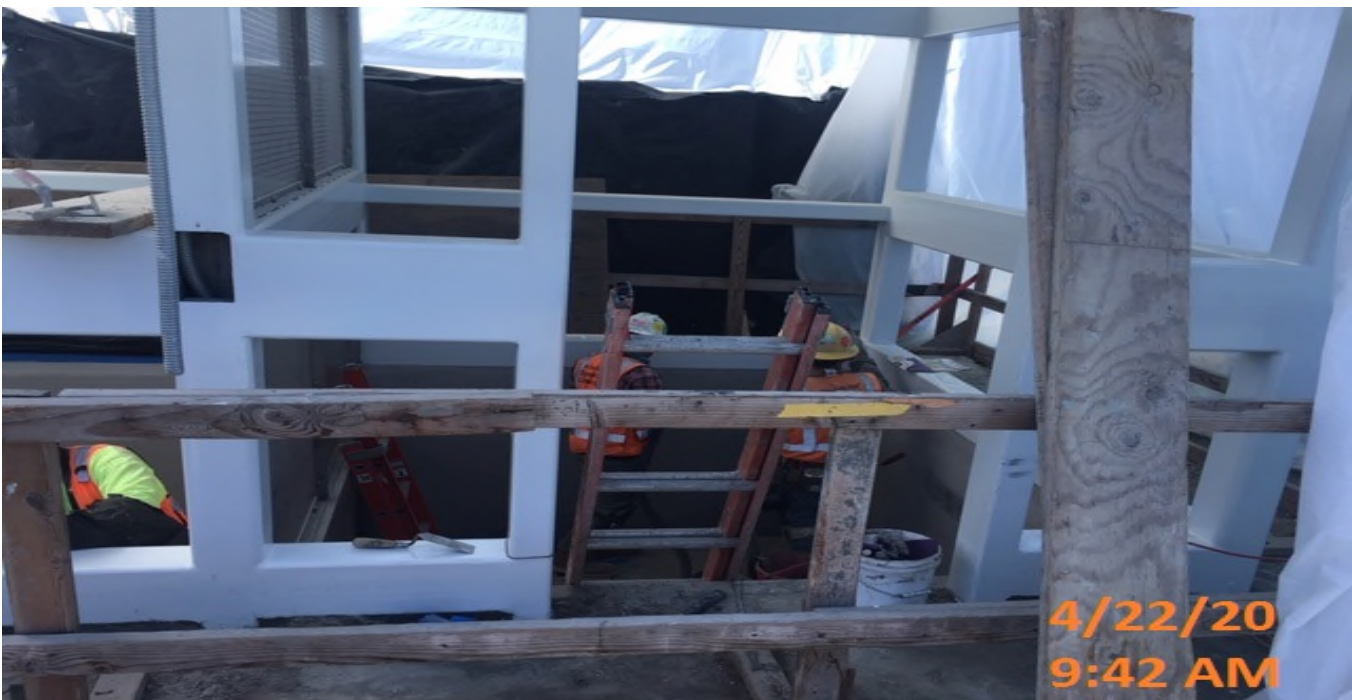
EXPO STATION – Continue patching and surfacing walls for Elevator shafts 1&2 at the plaza level.
