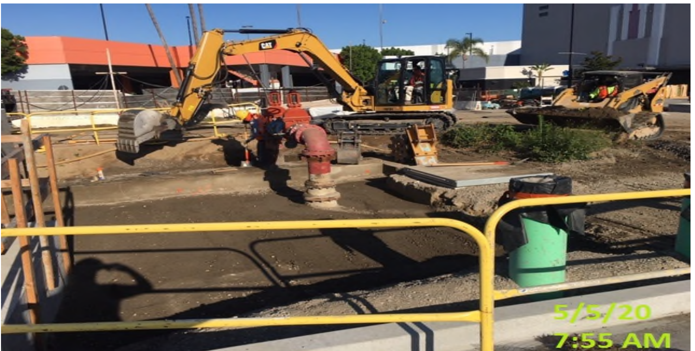
MLK STATION – Resume backfilling areas around the water backflow preventer valve on the east side of the plaza level.
