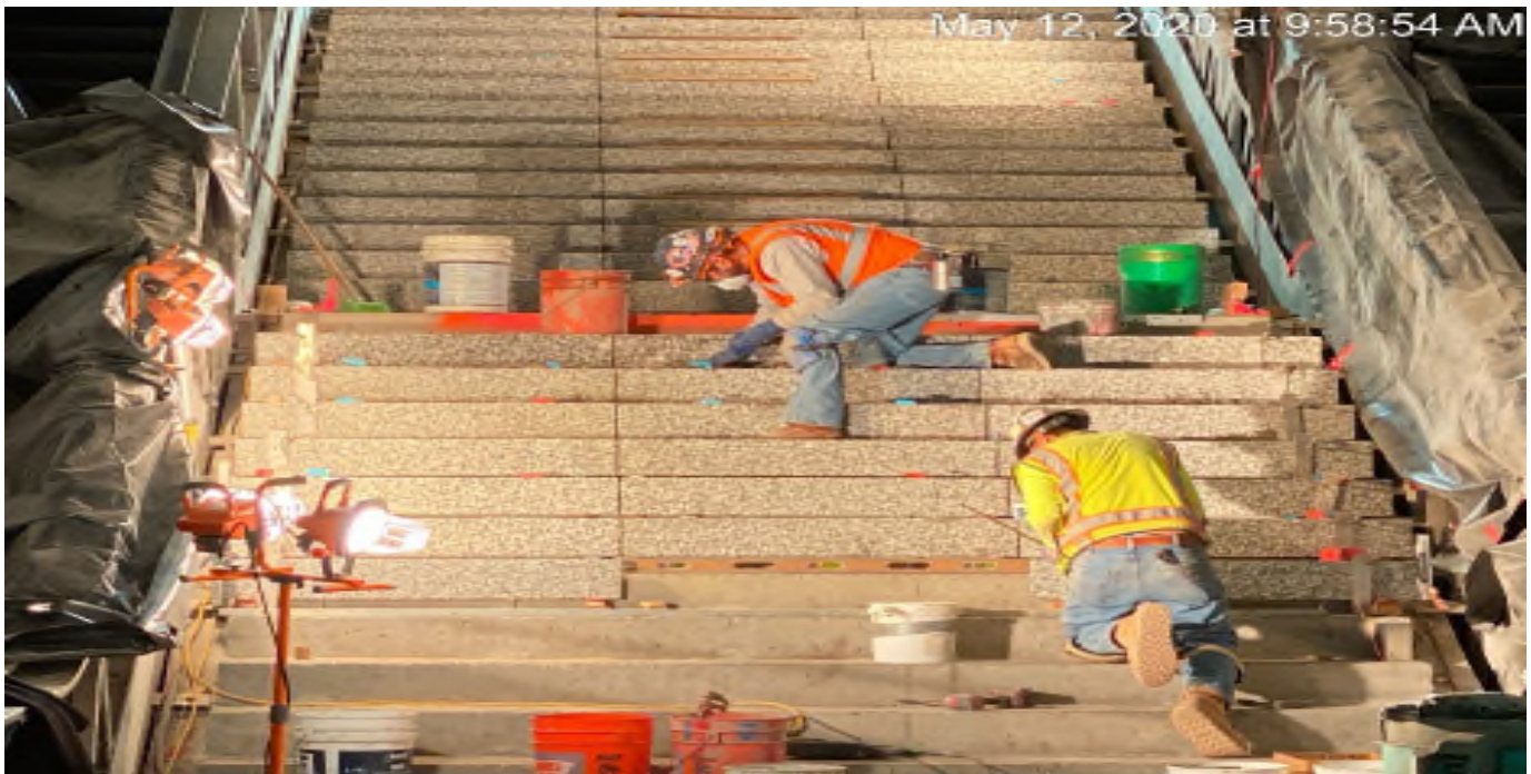
LEIMERT PARK STATION – Continue granite thread and riser installation at the intermediate stair case landing.
