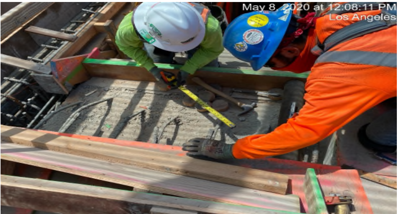
LEIMERT PARK STATION – Continue drilling and doweling for the north emergency exit hatch doors at the plaza level.
