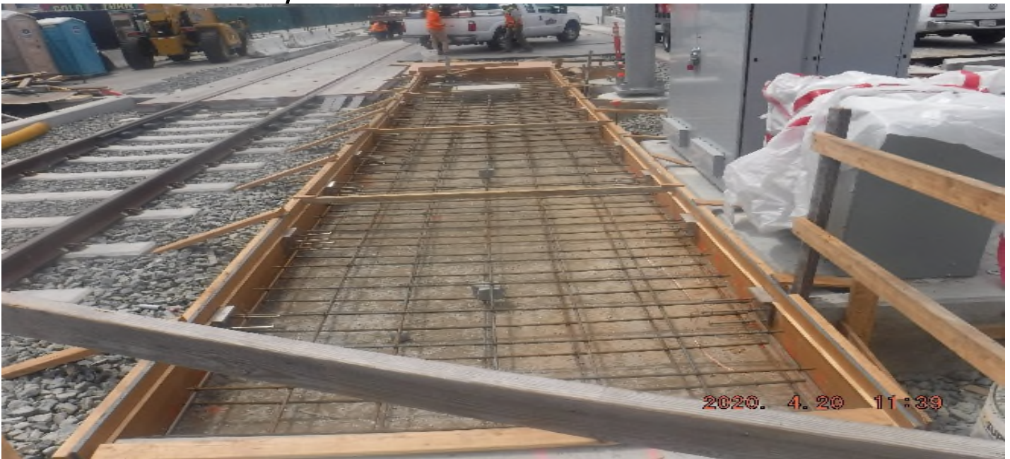
Crenshaw / Slauson - STA 323+00 TK#3/SB looking west – track structure disturbed (between tracks) north end of Slauson Station – PUNCH LIST
