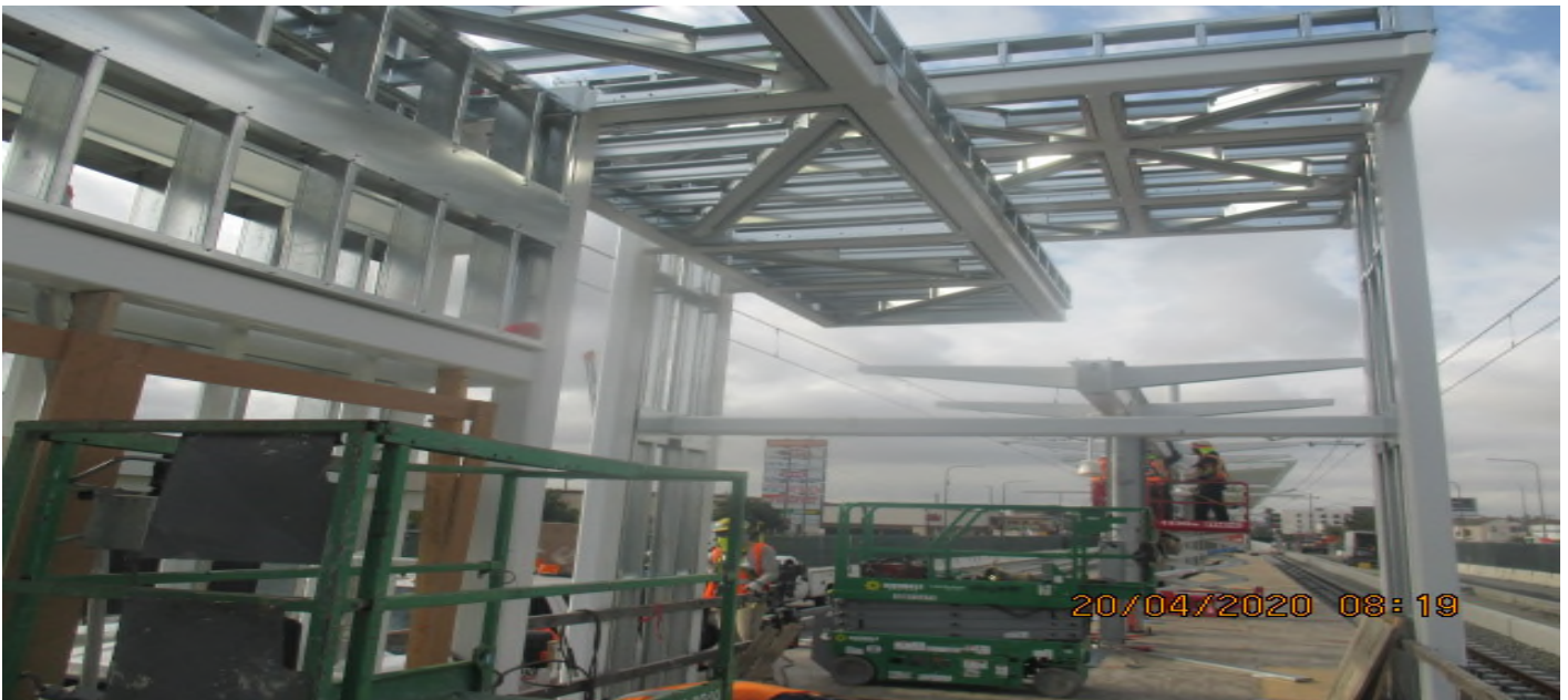
Hyde Park Station – Continue installing light gauge framing and roofing on the north end canopy structures. 4/20/20
