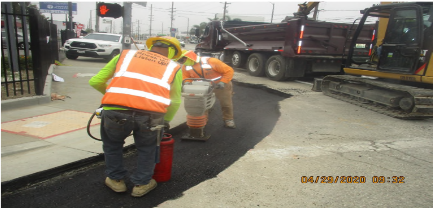
MANCHESTER STREET- WSCC Slot pace trench at N.E COR of Manchester and Florence.
