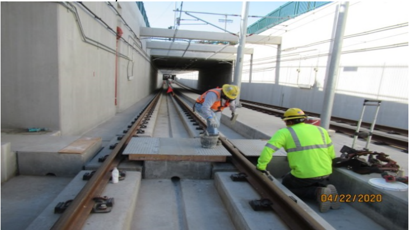
UG1 – WSCC repair work on emergency walkway crossing in UG1 SB #3 track STA 49+73
