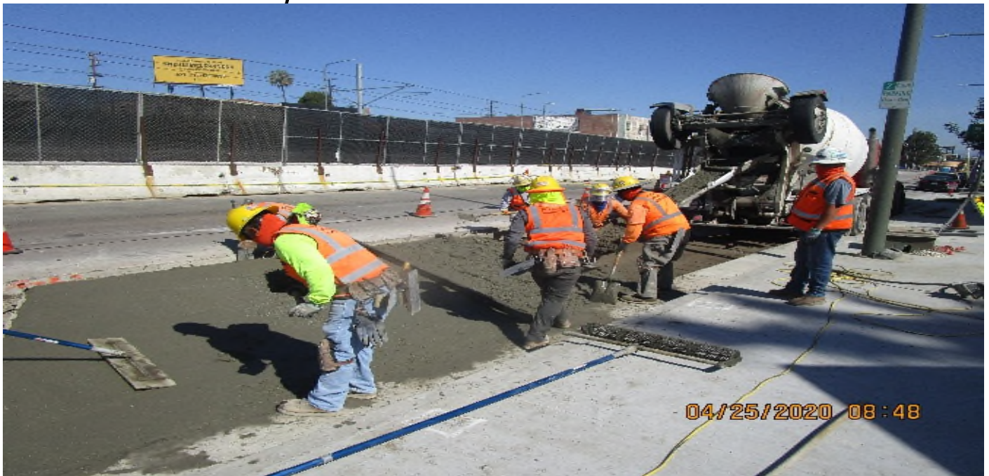
LEIMERT PARK STATION – Placing concrete for the new bus pad installation on the north east corner of 48th St and Crenshaw Blvd.
