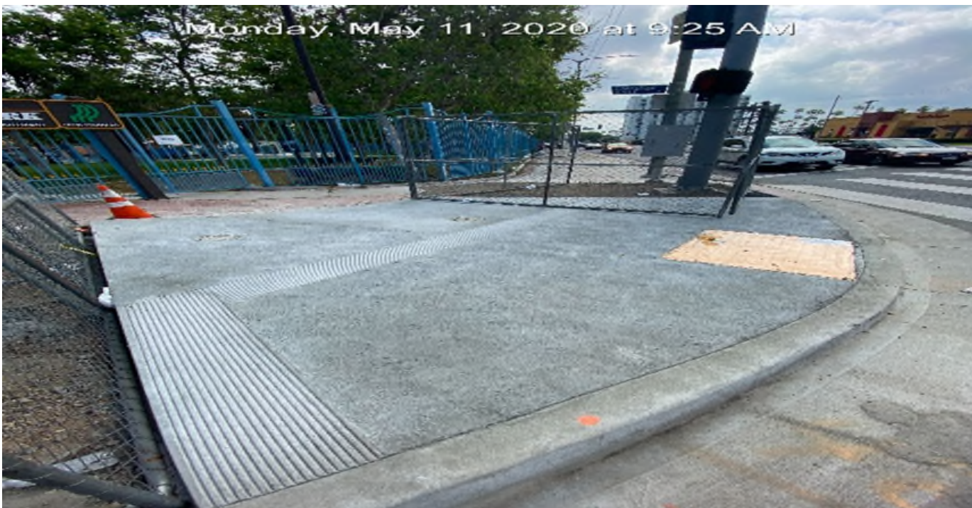
LEIMERT PARK STATION – Completed ADA ramp installation on the northeast corner of Vernon Ave and Crenshaw Blvd.
