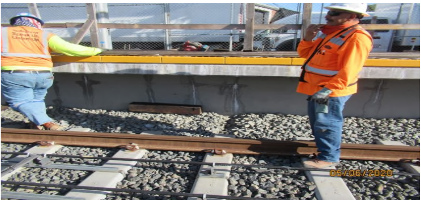
HINDRY STATION- WSCC removed ballast around treaded timber ties to level them equaling to Comon ties at Hindry station platform SB #3 track rework
