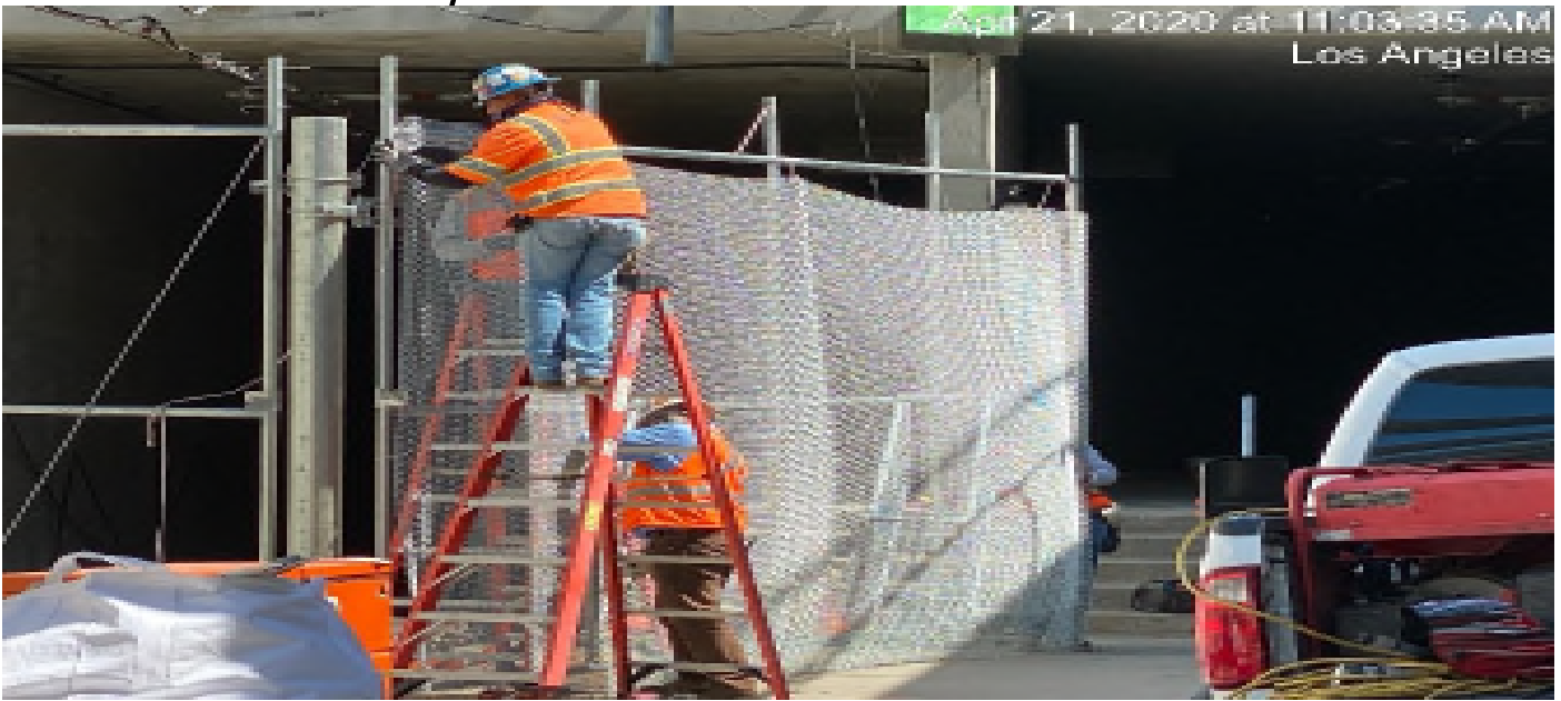
UG3 – Installing chain link fencing for both north and southbound tracks at the south end portal entrance.
