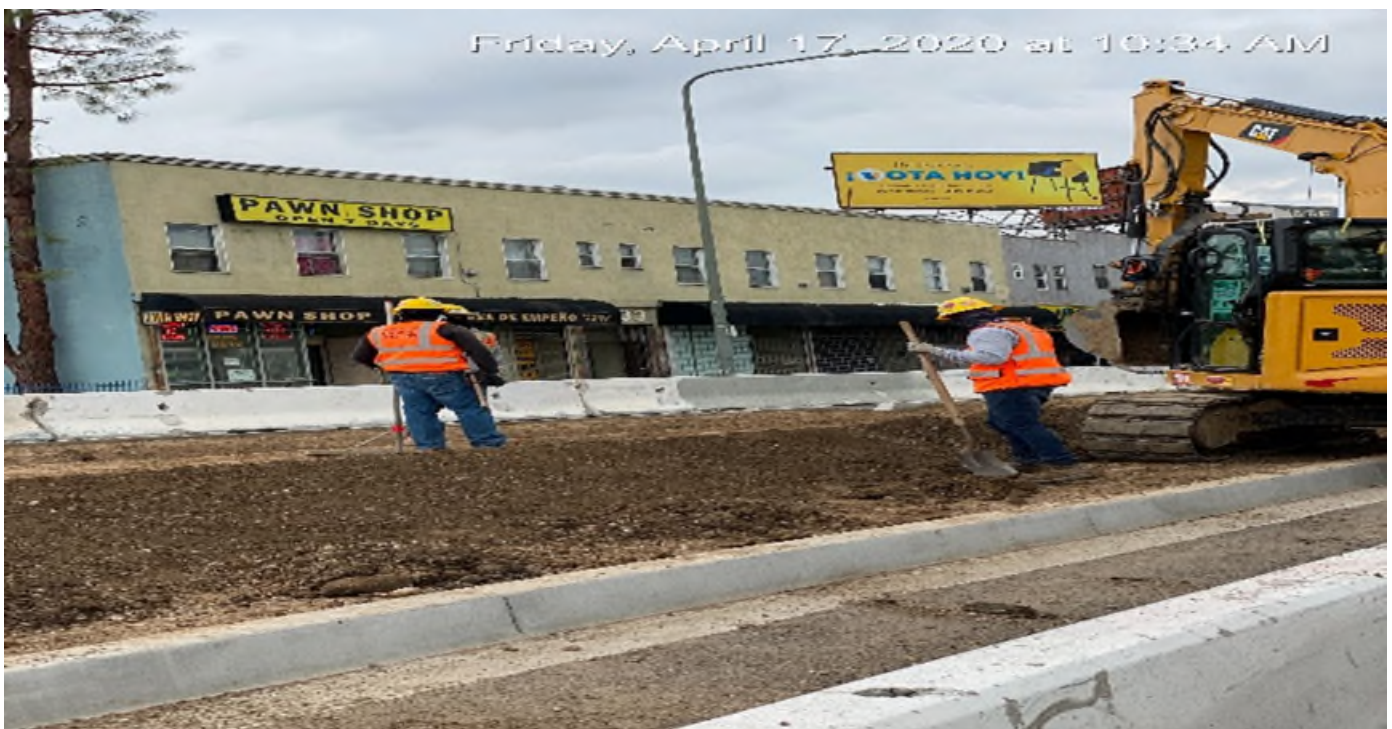
LEIMERT PARK STATION – Continue backfilling/grading the center guideway median island for drainage on Crenshaw Blvd between 48th St and Vernon Ave.
