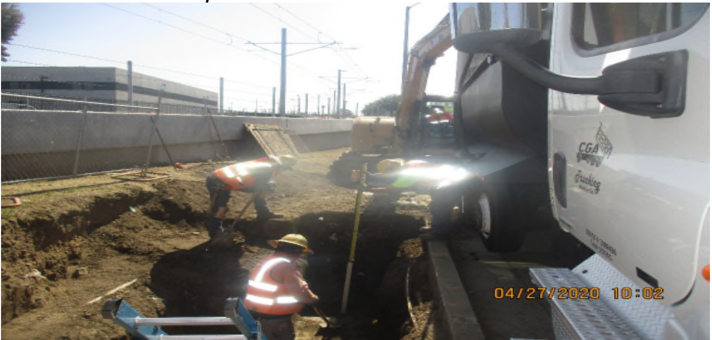
Florence/Brea – WSCC Excavate for CB west of La Brea on W/B Florence.
