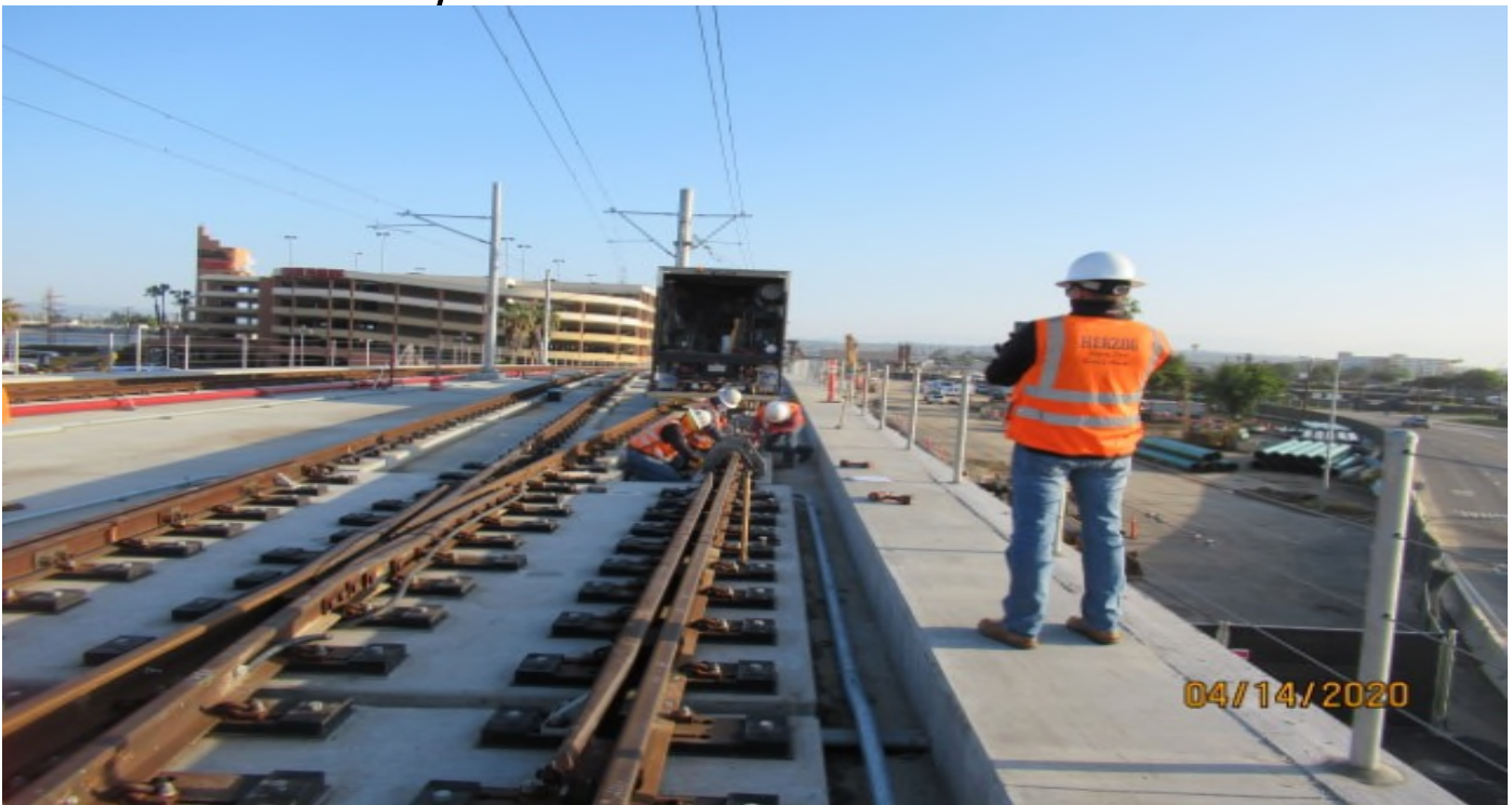
Aviation/Century – HCC, repairing cross levels on 10K1LH XO Century-Aviation Bridge NB # 4 track.
