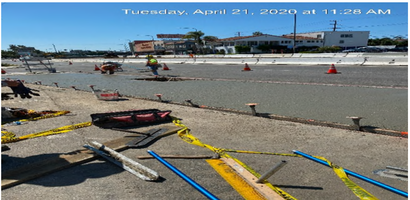
LEIMERT PARK STATION – Placing concrete for new sidewalk installation for the center “Pork Chop” median island on Crenshaw Blvd between 46th St and Leimert Blvd.
