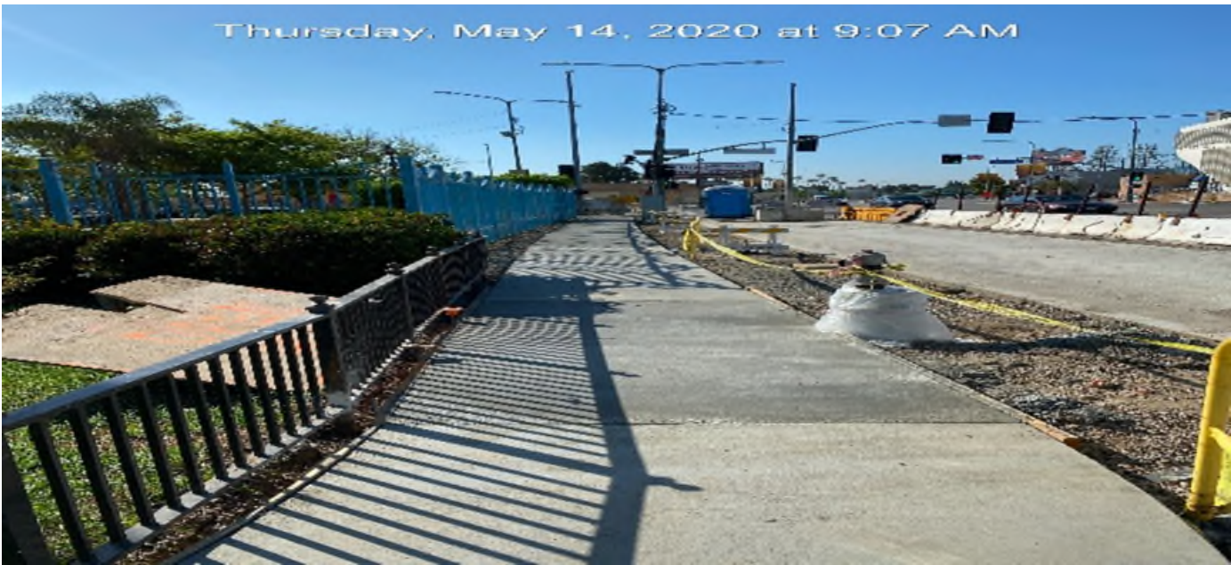
LEIMERT PARK STATION – Completed concrete placement along the northbound sidewalk on Crenshaw Blvd between Vernon Ave and 43rd Pl.
