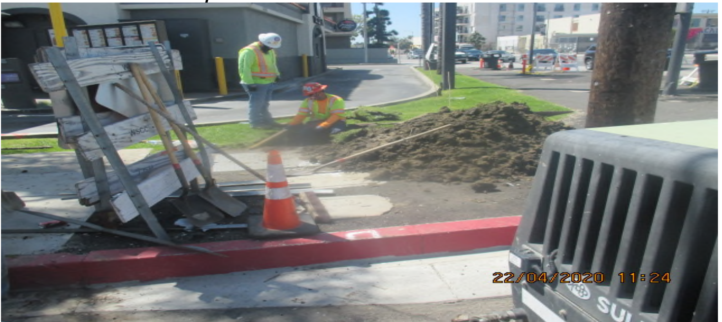
PARK MESA – Excavating for light pole foundations on the south east corner of 60th St & Crenshaw Blvd. 4/22/20
