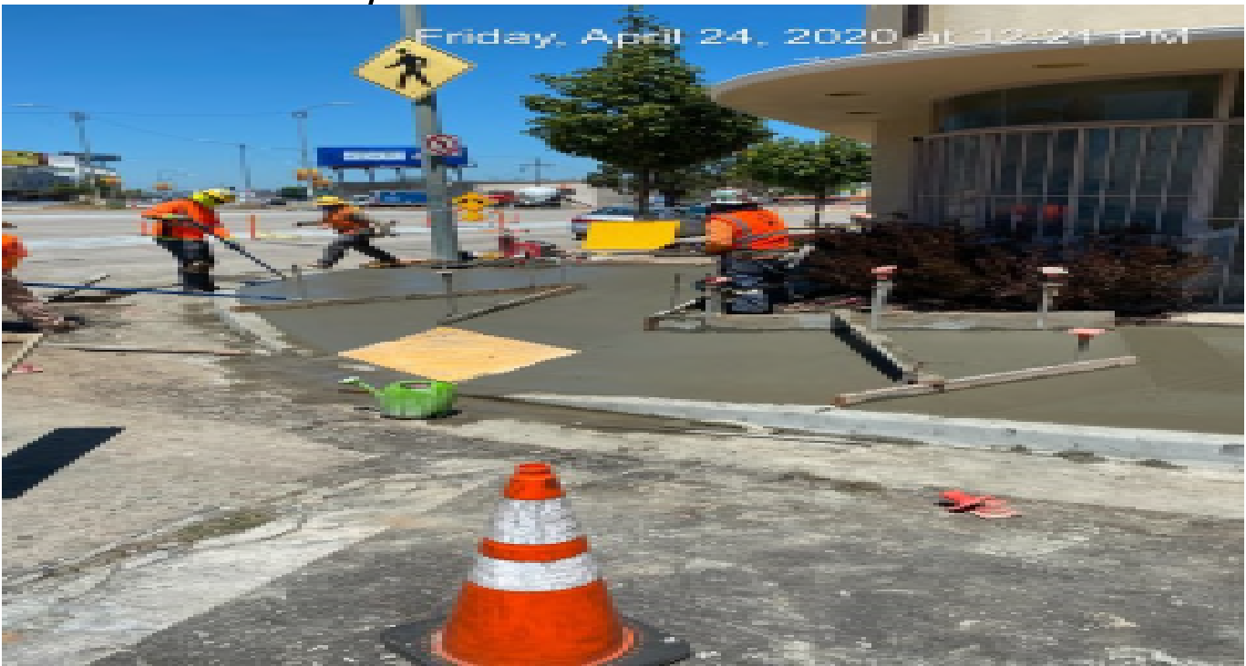
LEIMERT PARK STATION – Continued placing concrete for the new sidewalk and ADA ramp installation at the northeast corner of 46th St and Leimert Blvd.
