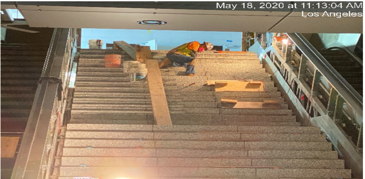
LEIMERT PARK STATION – Continue granite thread and riser installation at the concourse stair case landing.
