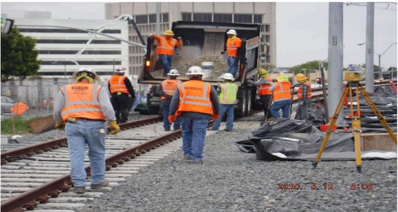
Florence/Brea - STA 206+00 TK#4/NB looking south – track ballast delivery south of La Brea Station
