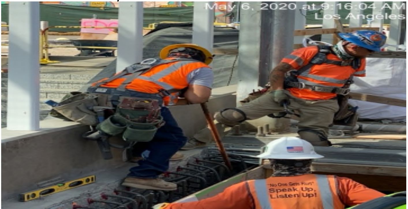
LEIMERT PARK STATION – Continue drilling and doweling for the north emergency exit hatch doors at the plaza level.
