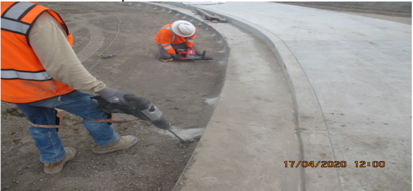
UG3 – Drilling and doweling the Cul-de-sac gutter radius at North Victoria Ave. 4/17/20
