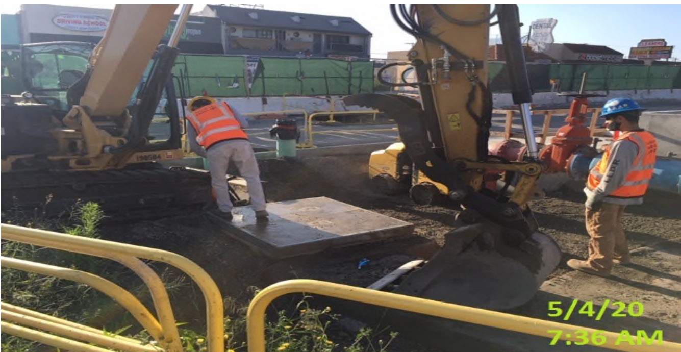
MLK STATION – Resume backfilling areas around the water backflow preventer valve on the east side of the plaza level.
