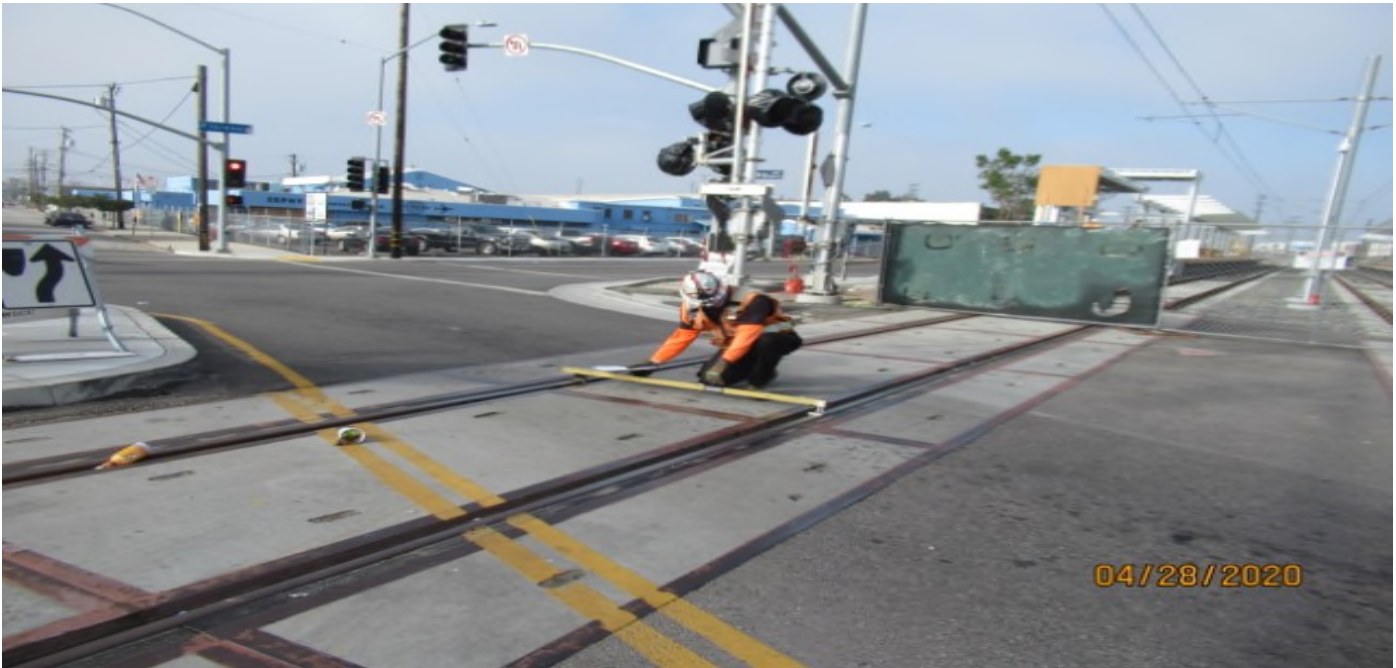
HINDRY STATION- WSCC QC track inspector verifying cross level on #4 NB track at Hindry grade crossing for BIM360 internal punch list updates (looking southeast)
