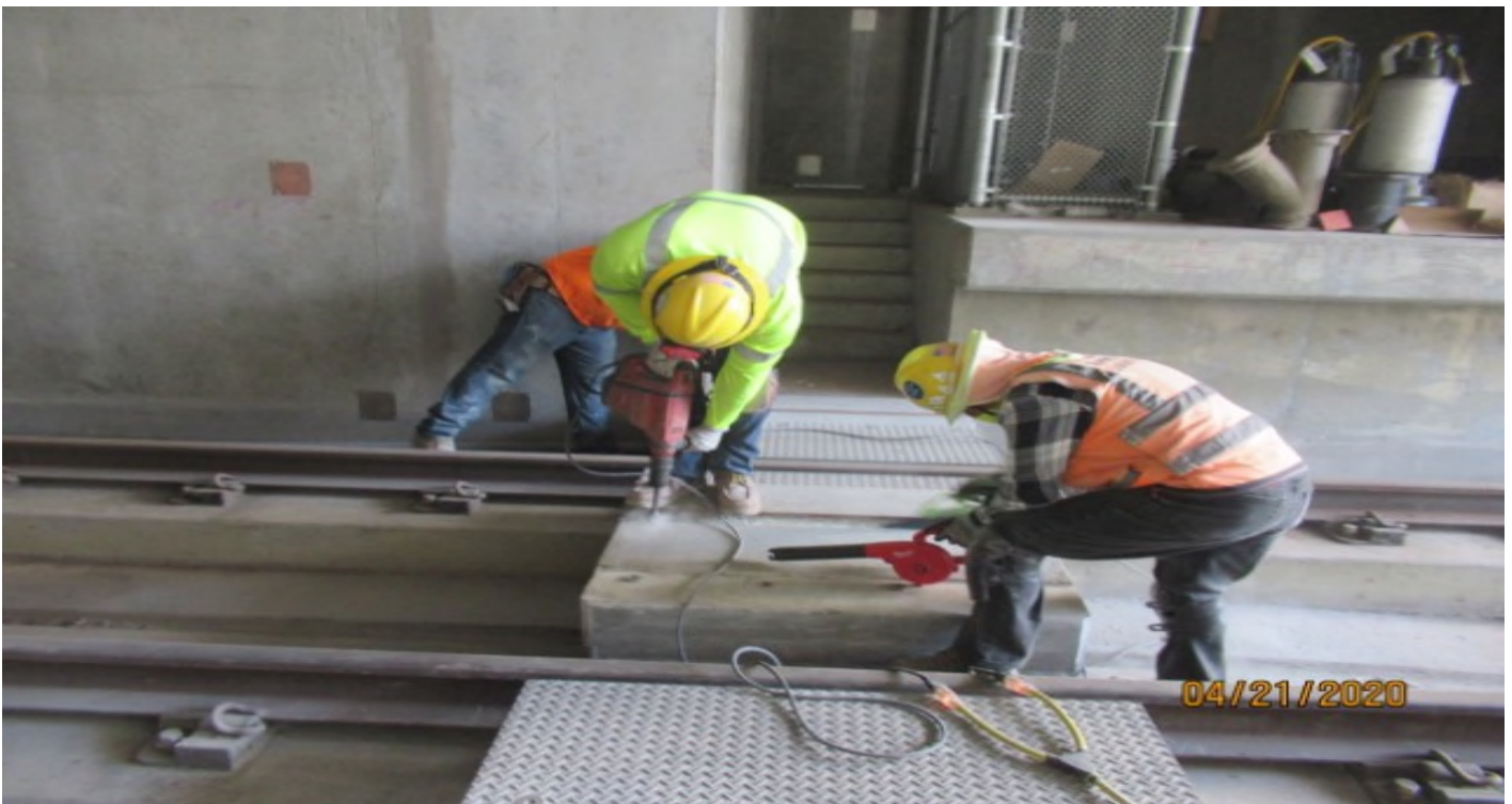
UG1 - WSCC repair work on emergency walkway crossing in UG1 SB #3 track STA 49+73.
