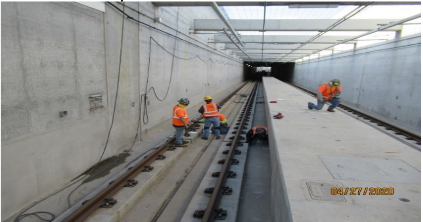
UG1 – WSCC installing epoxy into expansion joints in UG1 NB #4 track (looking south) out of sequence
