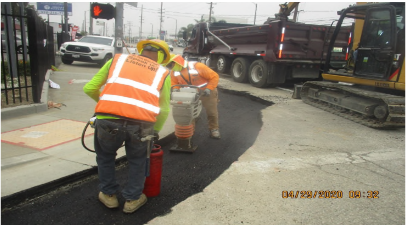
Manchester Bridge – WSCC Slot pace trench at N/E CORNER of Manchester and Florence.
