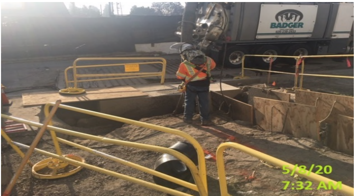
MLK STATION – Continue trenching and potholing for 12” HDPE drainage pipe system at the northern section of the plaza level.
