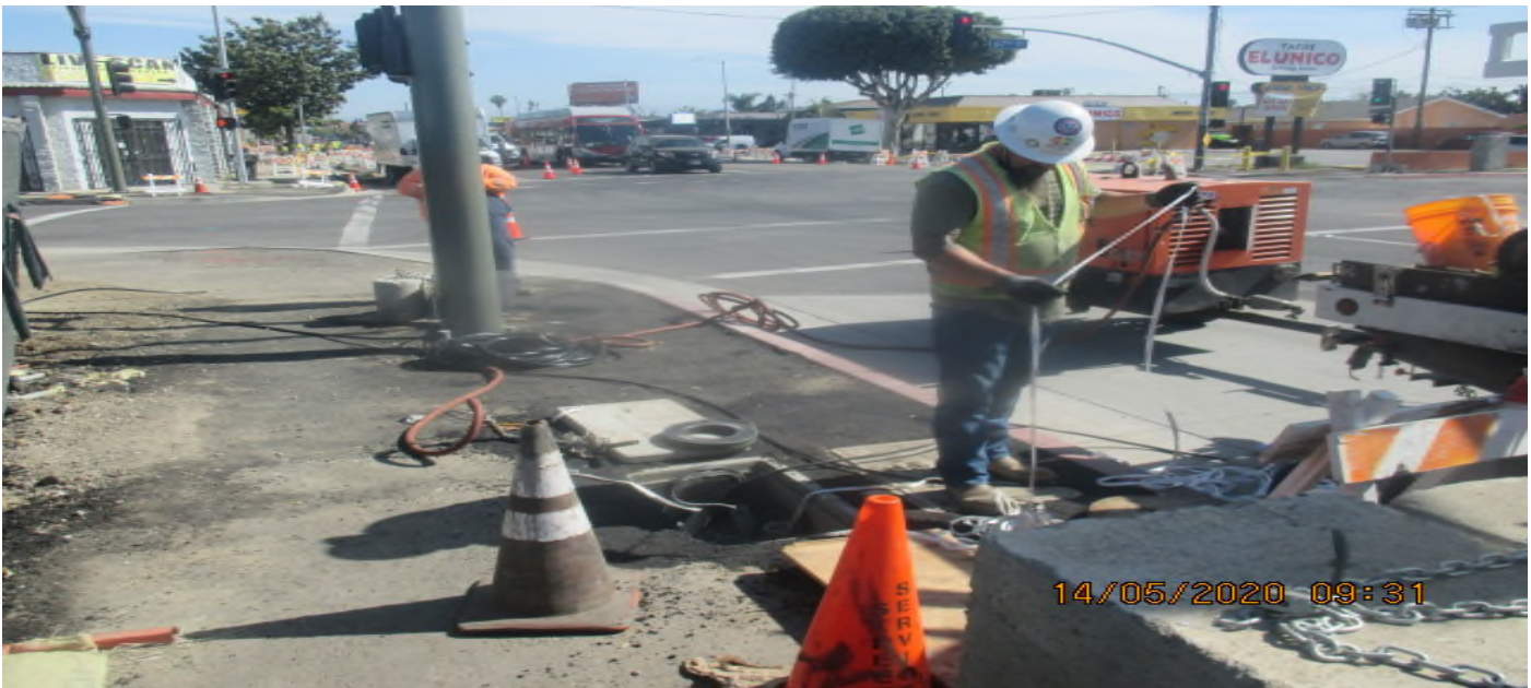
UG3 – Pulling power to pull boxes to supply runs for the street light pole on the southwest corner of 67th St and Crenshaw Blvd. 5/14/20
