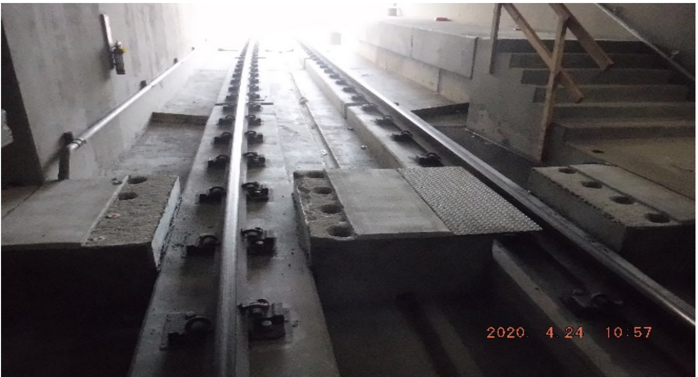
UG-4- STA 371+65 TK#4/NB looking south – steel plates and inserts removal at crosswalk UG4 – PUNCH LIST
