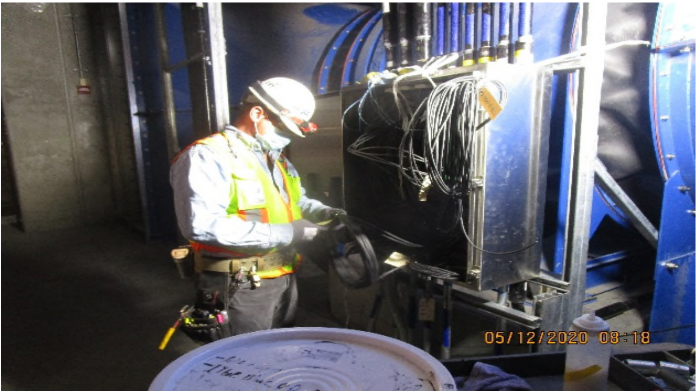
Crenshaw/Vernon - Vernon Concourse, Emergency fan room pulling #14 # Type RHW-2 wire (EVF-302) to TFD-6-302 (PWR) limit switches
