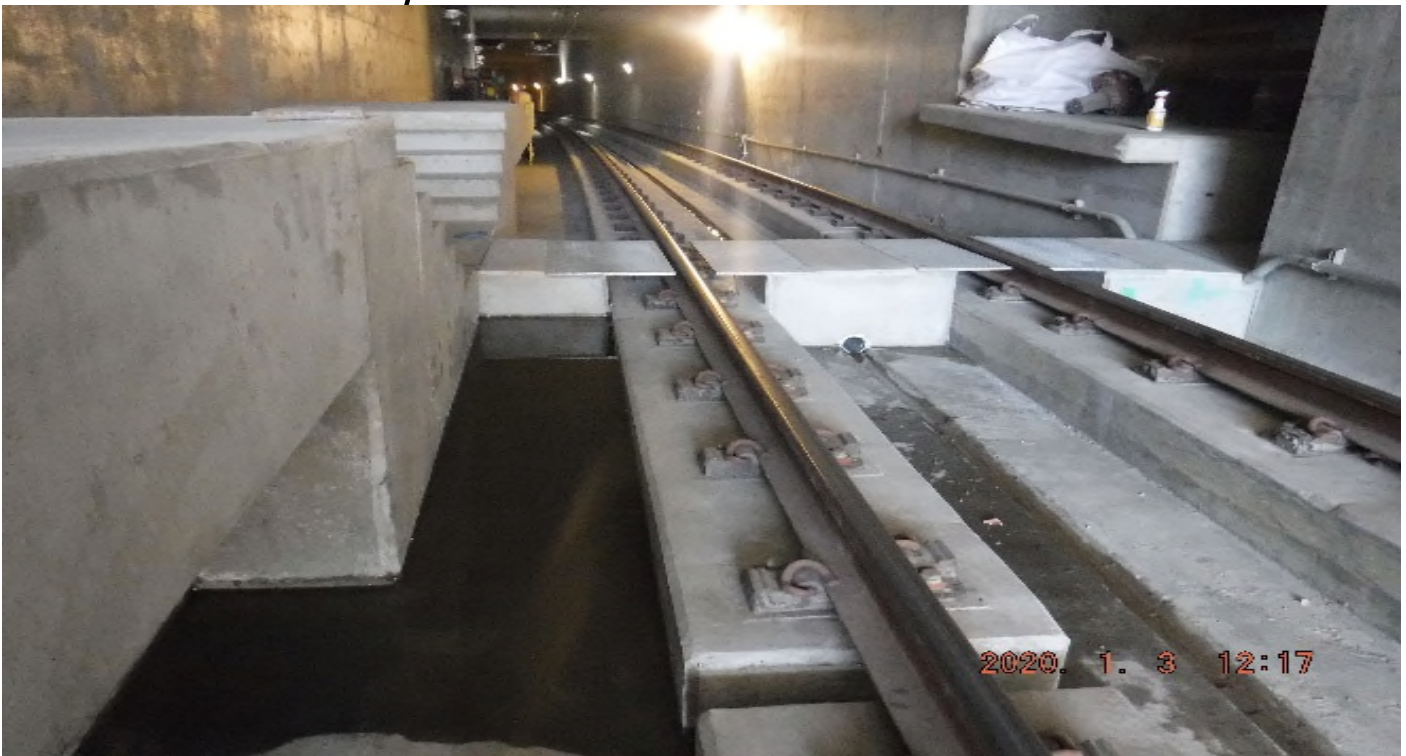
UG-4- STA 371+65 TK#4/NB looking north – steel plates set at crosswalk UG4 at the end of 2019 – PUNCH LIST
