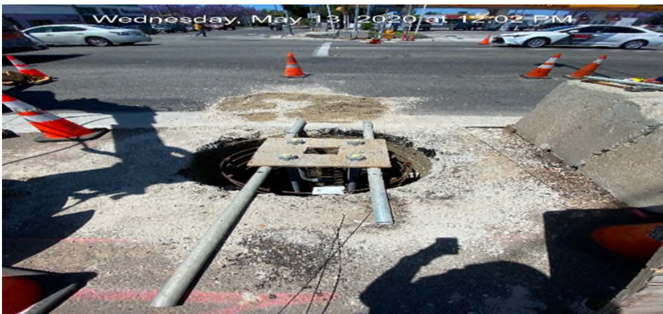
EXPO STATION – Excavating and installing rebar for the street light foundation on the northeast corner of Obama Blvd and Crenshaw Blvd.
