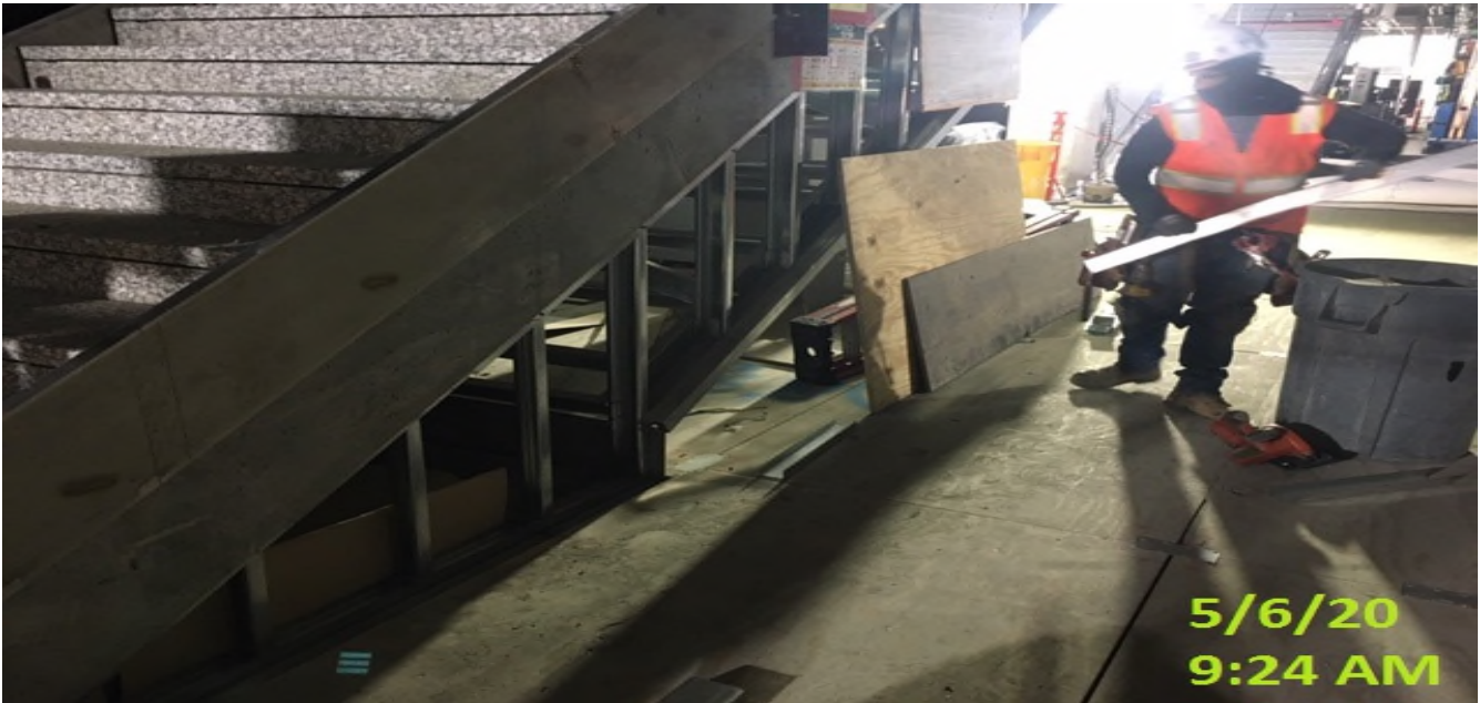
EXPO STATION – Installing metal steel framing at the underside of escalators 3&4 and stairwells 2&3 at the platform level.
