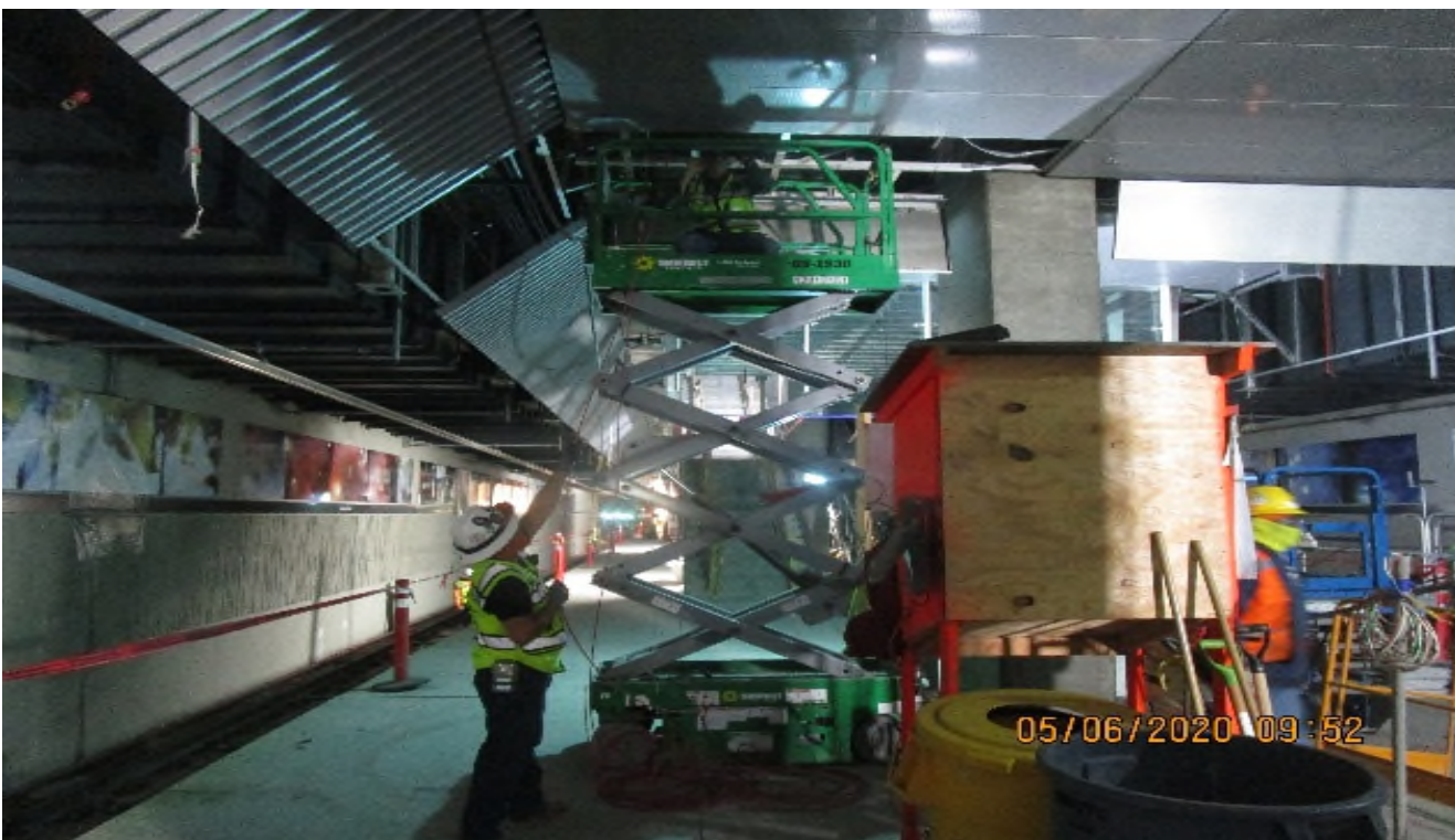
Crenshaw/Vernon - Vernon North Platform, continued begin pulling smoke detector 1 pair #18 from devices to Electric (N) T115
