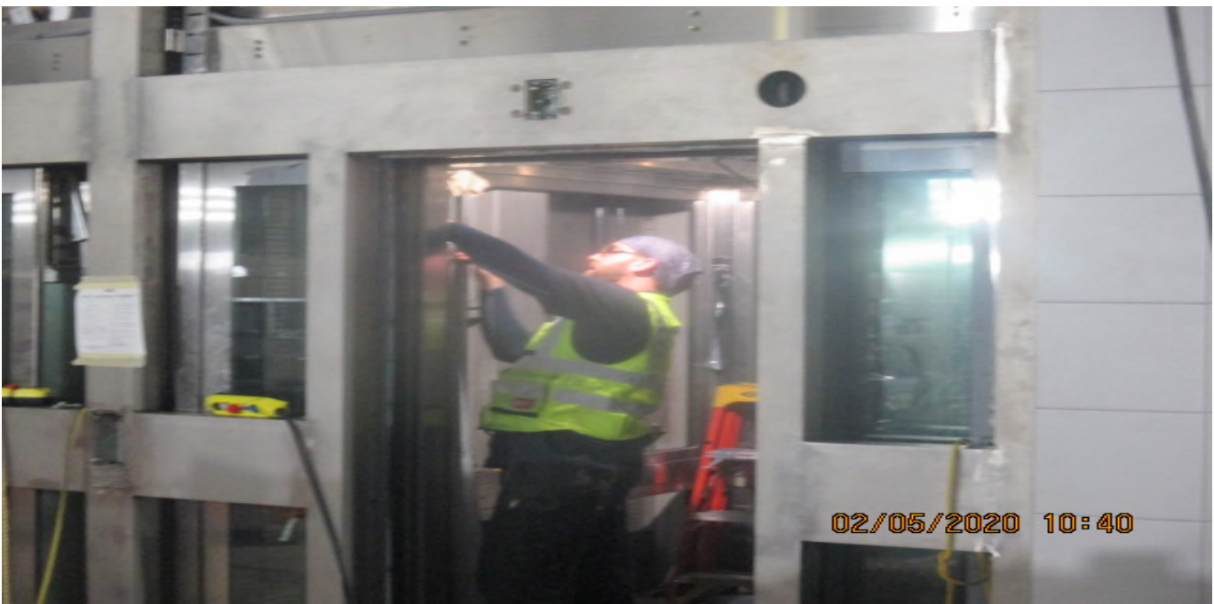
LEIMERT PARK STATION – Wiring and adjusting elevator cabs 3&4 at the concourse level. 5/2/20
