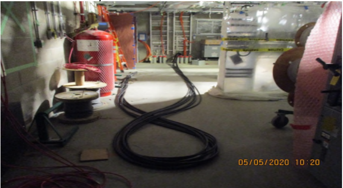
MLK - Train Control Cable Pulled in the TC&C Room, MLK Station, Looking North
