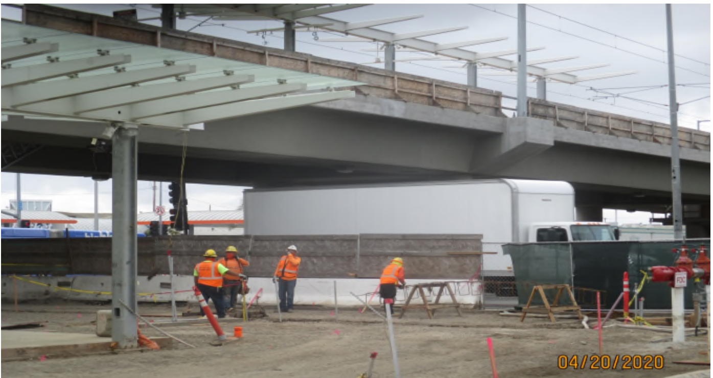
Aviation/Century - Building a rebar cage for the bollards at the Aviation Station.
