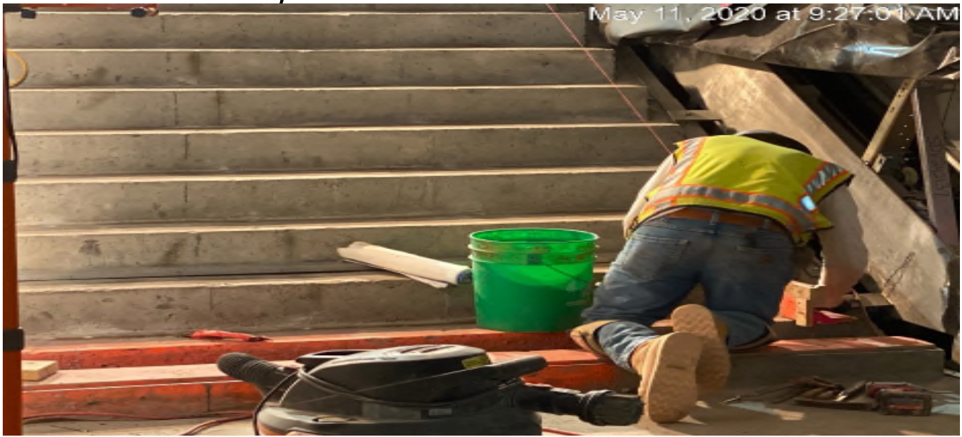
LEIMERT PARK STATION – Continue granite thread and riser installation at the intermediate stair case landing.
