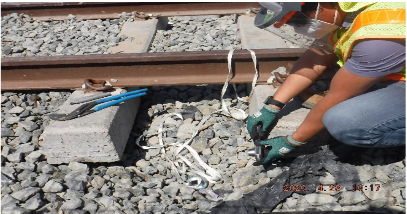
57 th Street - STA 329+90 TK#4/NB looking west – checking depth of system conduit imbedded in track structure south of 57th St.
