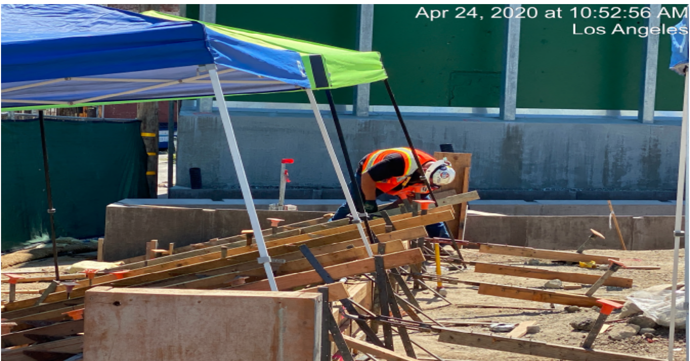
LEIMERT PARK STATION – Continue formwork for the planter stair risers on the northwest section of the plaza level.
