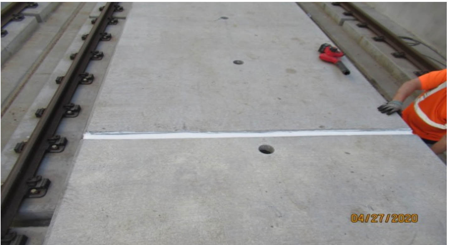
UG1 – UG1 SB #3 track STA 49+78 emergency walkway on-going repair work (looking west) Rework
