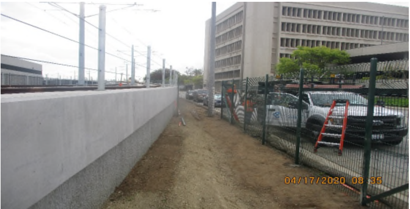
Florence/Ivy – ACE Fence Placed fence panels at Florence east of Ivy crossing.
