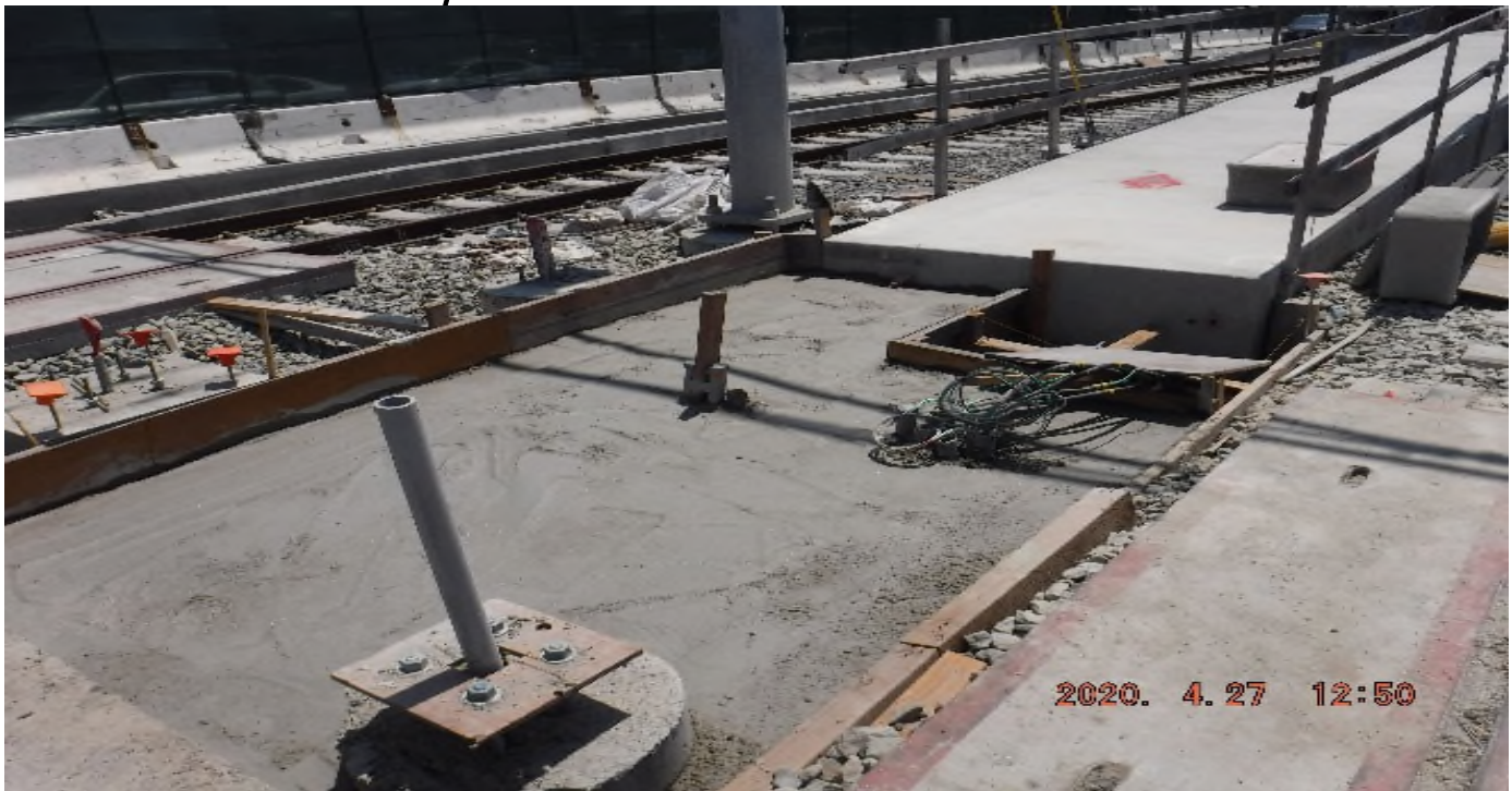
Crenshaw / Slauson - STA 323+00 TK#3/SB looking south – set form and rebar at north end of Slauson Station for future pedestrian pad
