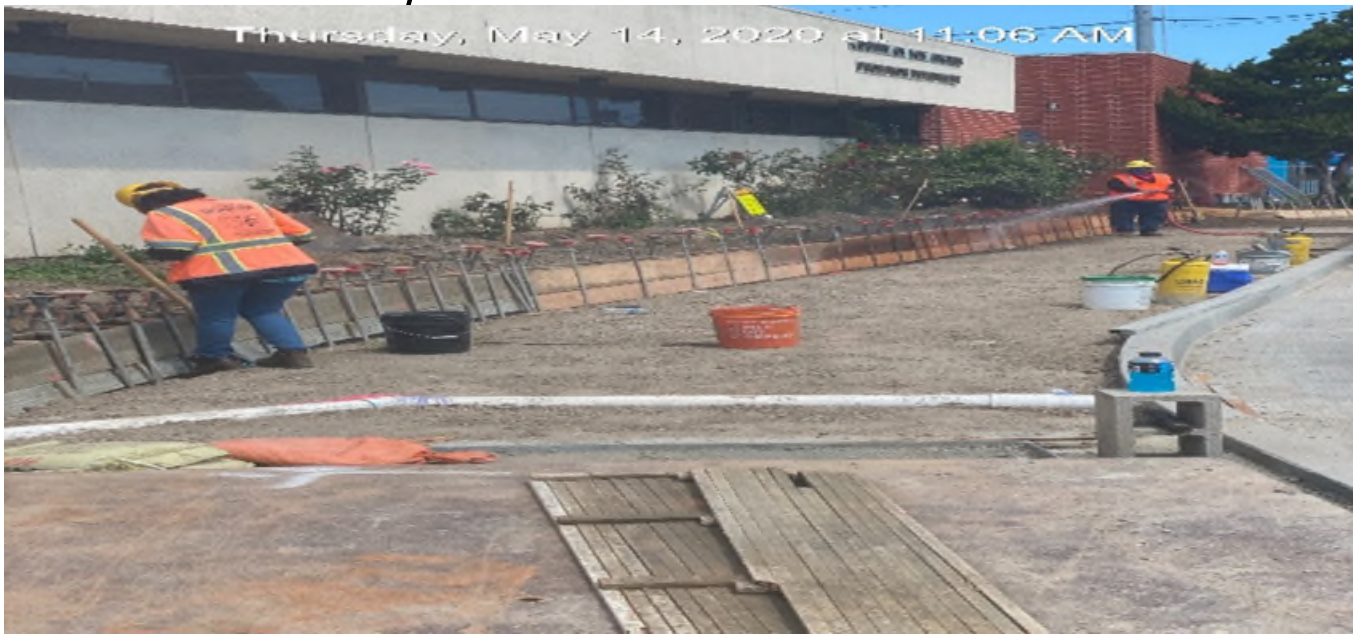
EXPO STATION – Preparing area for concrete placement of sidewalk/curb installation on southbound Crenshaw Blvd between Exposition Blvd and Rodeo Blvd.
