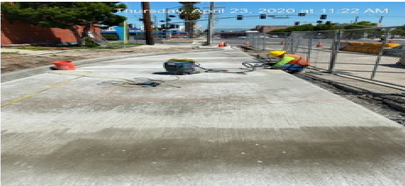
EXPO STATION – Stripping forms and saw cutting the bus pad on southbound Crenshaw Blvd between Exposition Blvd and Rodeo Blvd.
