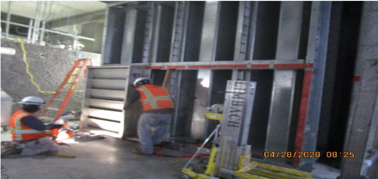
MLK STATION – Continue bird screen protection and hardware support to TFD-7-121 in the South Tunnel Vent Plenum C – 103 of the concourse level.
