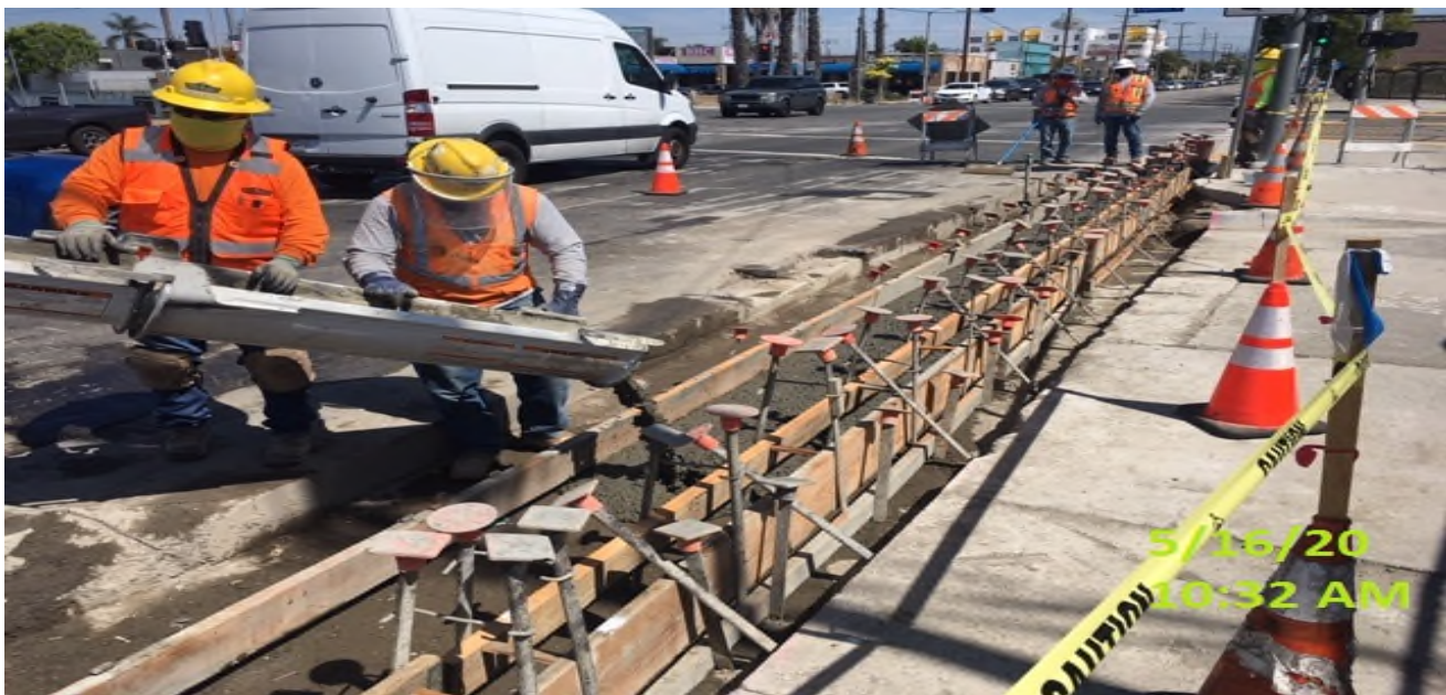
EXPO STATION – Placing concrete for new curb/gutter installation on northbound Crenshaw Blvd between Obama Blvd and Exposition Blvd.
