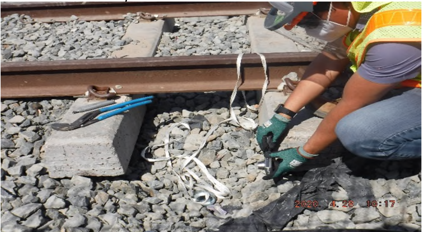
57th STREET- STA 329+90 TK#4 , NB looking west – checking depth of system conduit imbedded in track structure south of 57th St – PUNCH LIST
