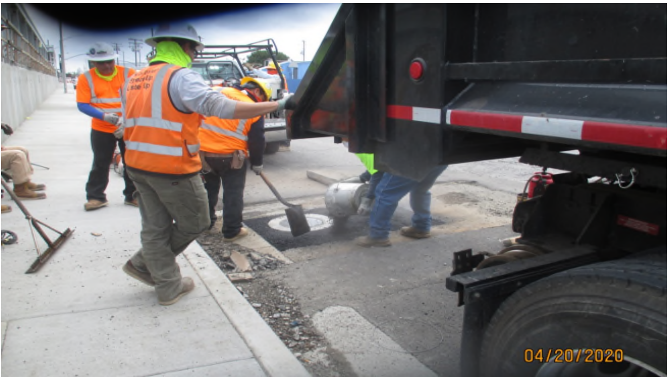
HINDRY STATION- AC being placed around the Hindry Station sump pump cleanout on Florence.
