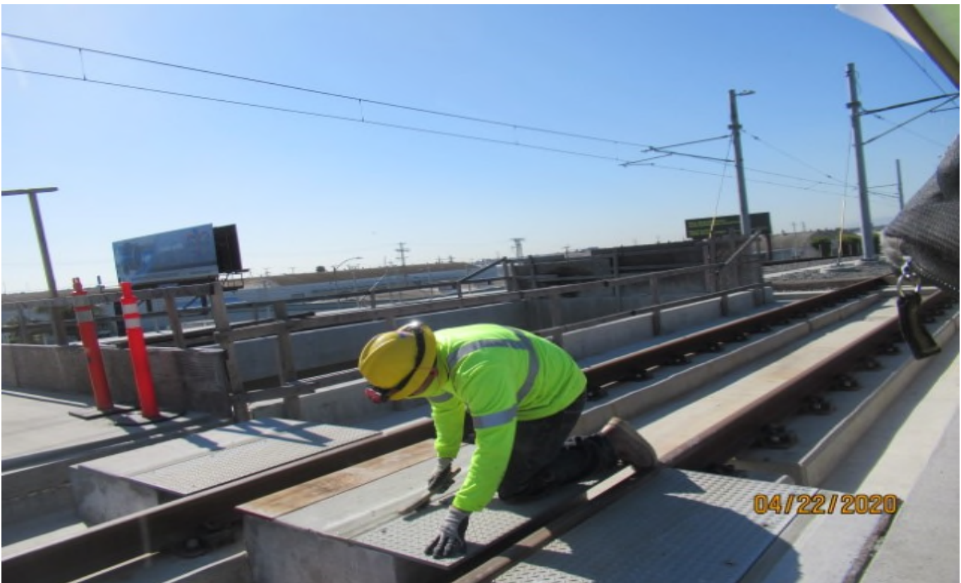
Aviation/Century – WSCC finalizing elevations on grout for emergency walkway crossing on SB #3 track STA 66+16 (looking southeast) Rework
