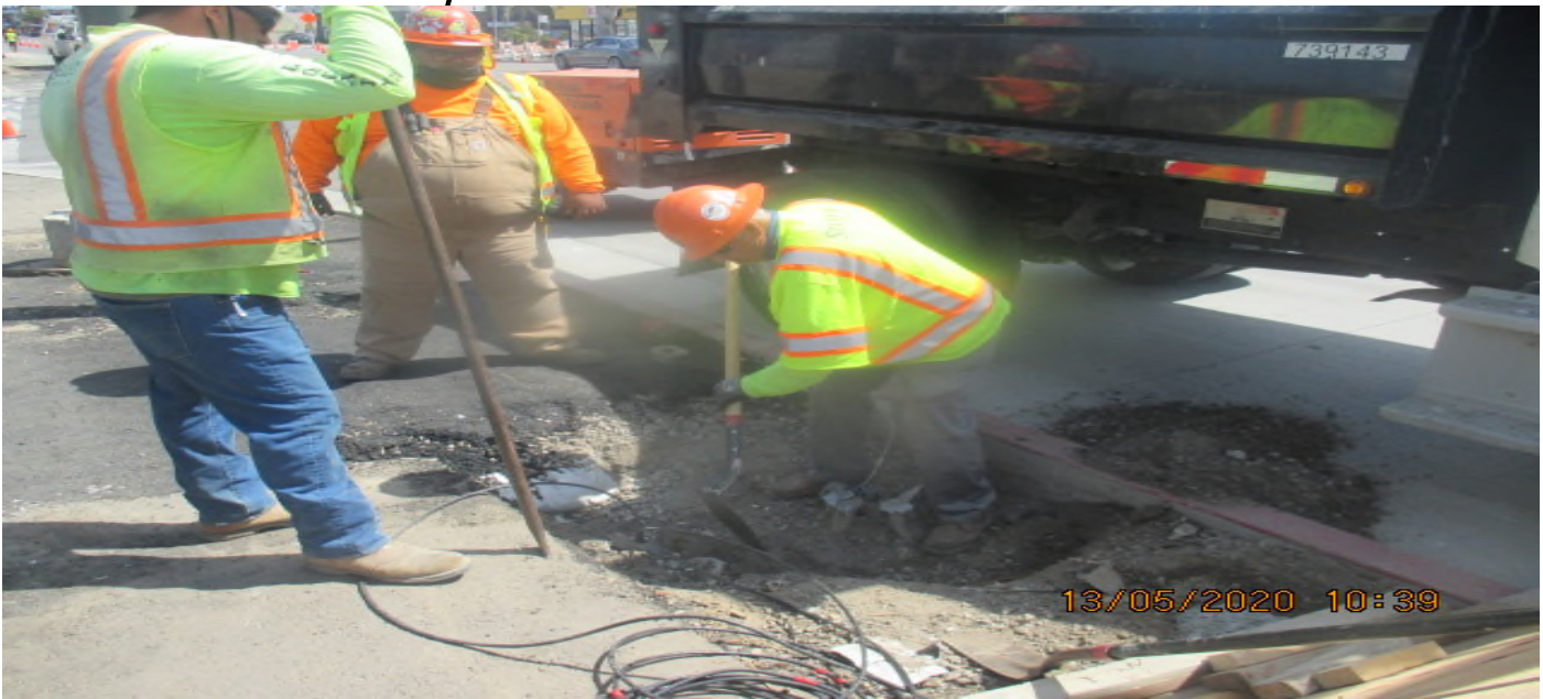
UG3 – Installing pull boxes for the street light pole on the southwest corner of 67th St and Crenshaw Blvd. 5/13/20
