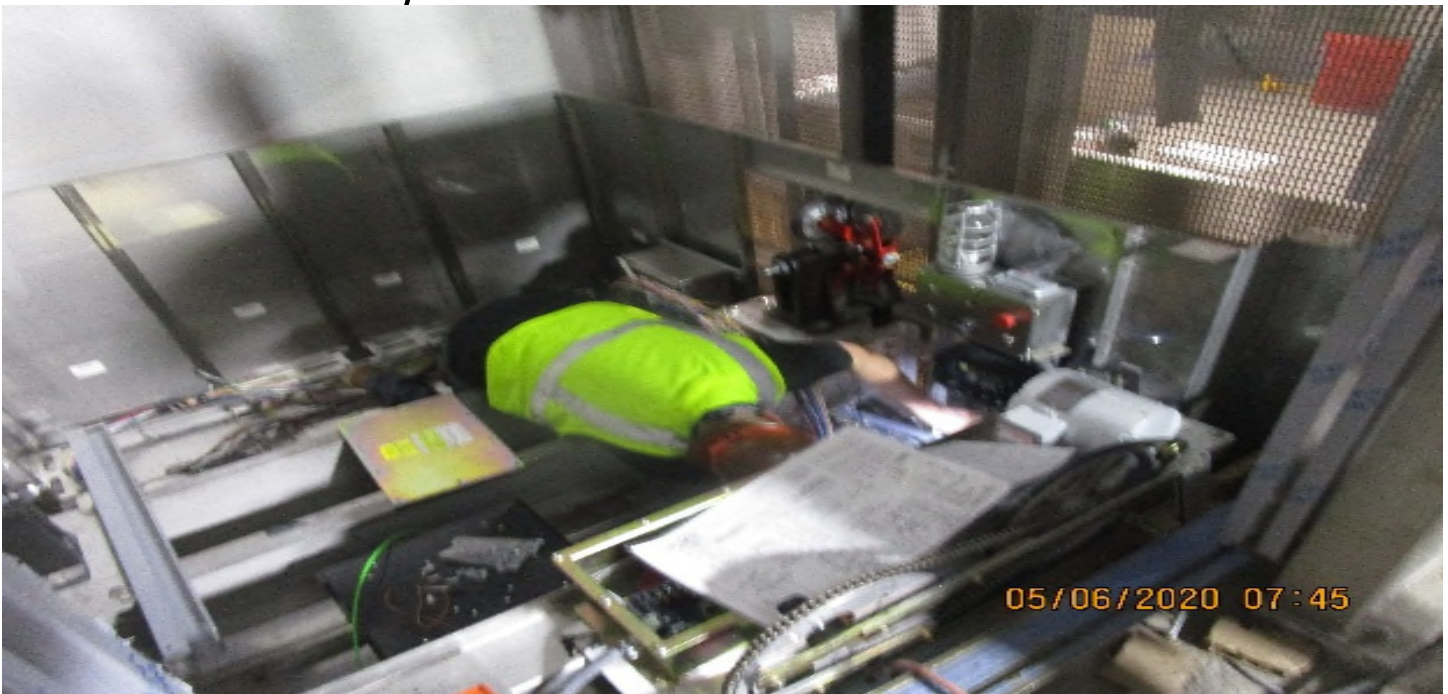
LEIMERT PARK STATION – Pulling/identifying wiring for switches/buttons for Elevators 1&2 at the concourse level.
