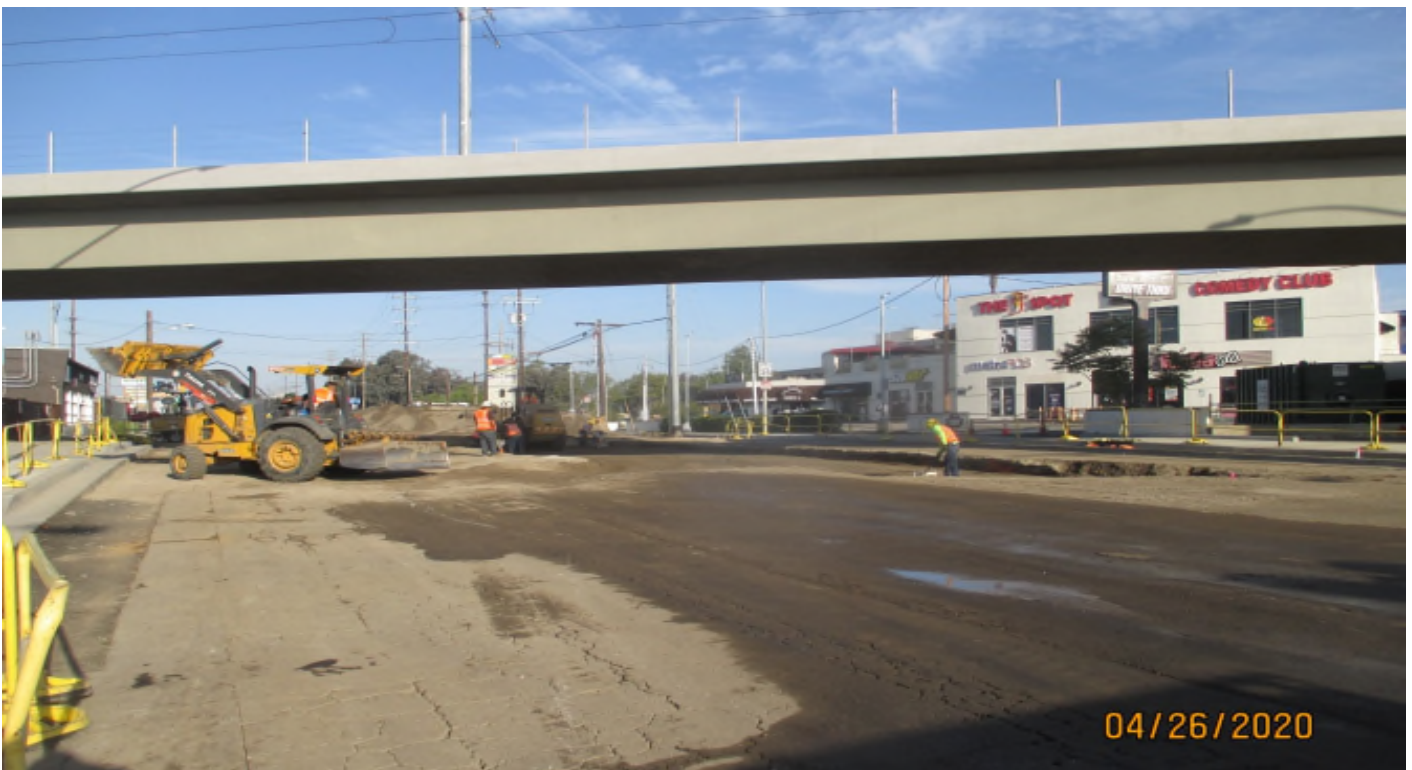
Manchester Bridge – Compaction of the base for the median and #1 WB lane on Manchester.
