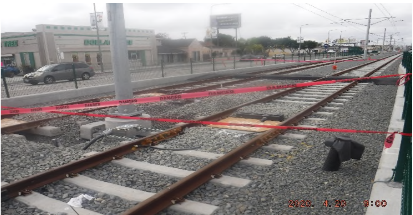
57 th Street - STA 330+00 TK#3/SB looking south – system work with track structure disturbance south of 57th St around/next to OCS #1258 as of 4.20.2020 – PUNCH LIST
