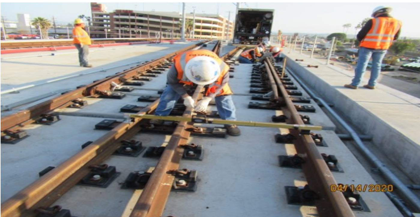
Aviation/Century – HCC installing Shim plates on 10K1LH XO on Century-Aviation bridge NB #4 track STA 70+50 (looking north) Rework
