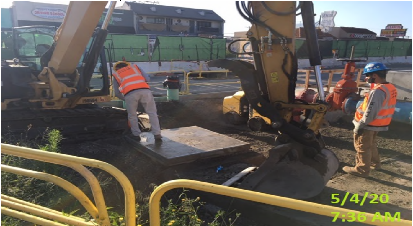
MLK Station - MLK – WSCC crew back filling area surrounding back flow valve
