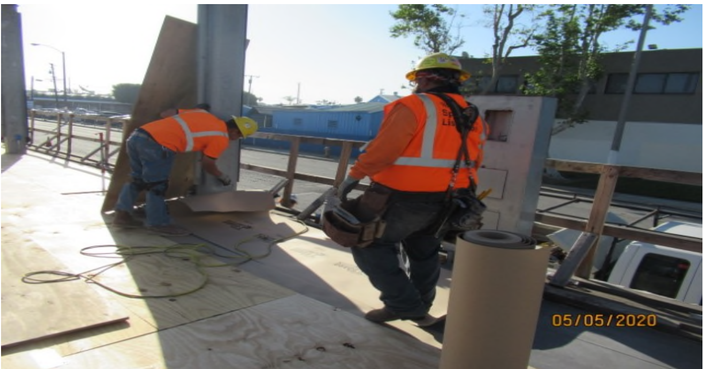
HINDRY STATION- WSCC installing protective plywood sheets onto newly placed colored concrete NB #4 Hindry station platform (looking northeast)
