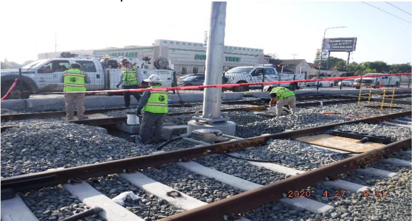
57th STREET- STA 330+00 TK#3,SB looking south (east) – system work with track structure disturbance south of 57th St around,next to OCS #1258 and MH-S099 – PUNCH LIST
