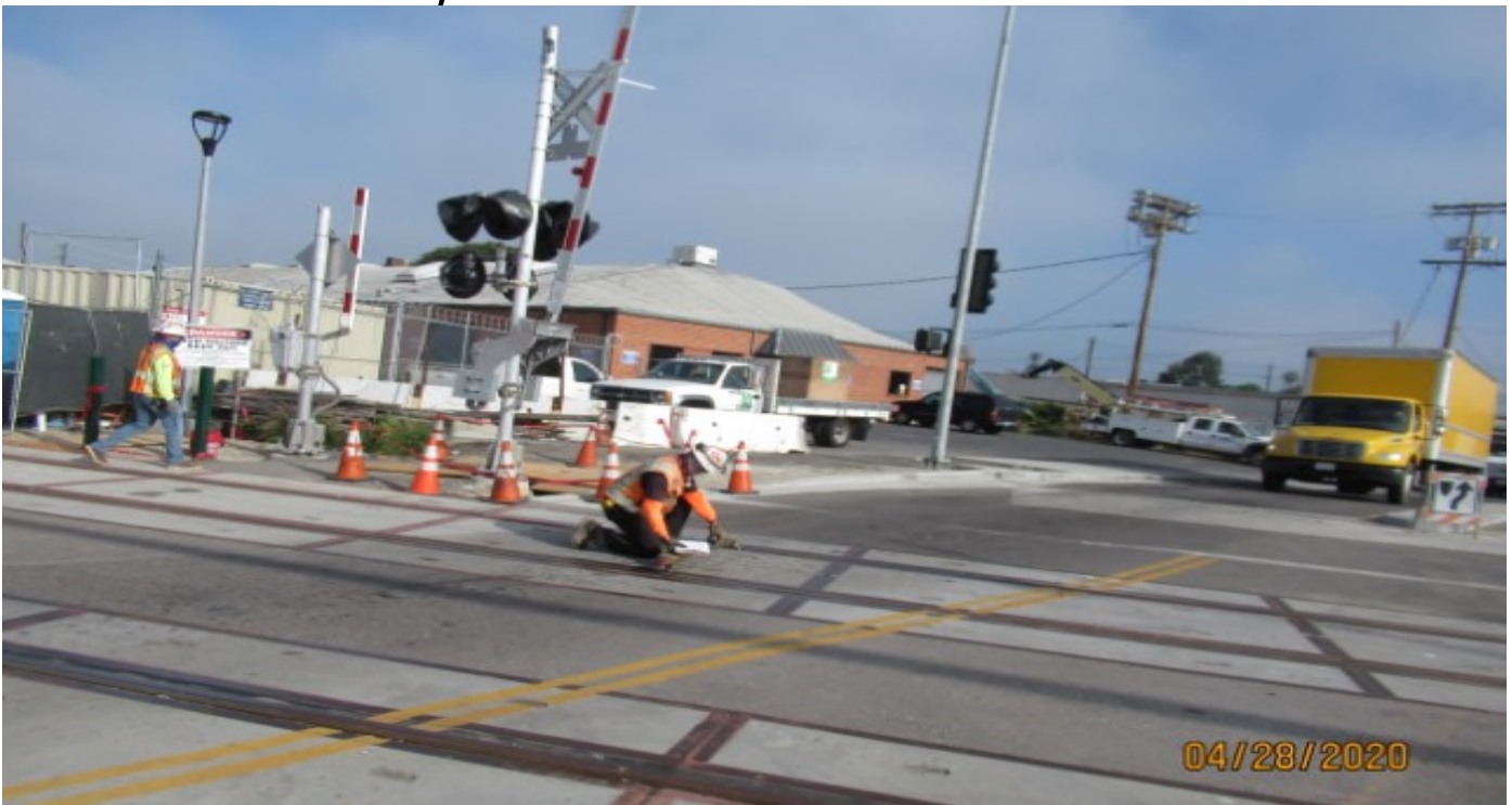
Florence/Hindry – WSCC QC track inspector verifying cross level on #3 NB track at Hindry grade crossing for BIM360 inturnal punch list updates (looking southeast)
