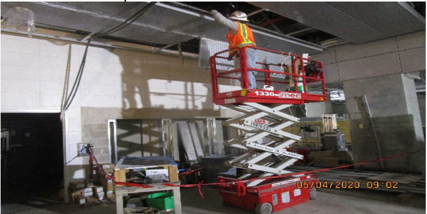
LEIMERT PARK STATION – Continue installing ceiling light fixtures at the concourse level.
