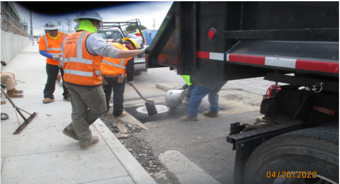
Florence/Hindry – AC being placed around the Hindry Station sump pump cleanout on Florence.
