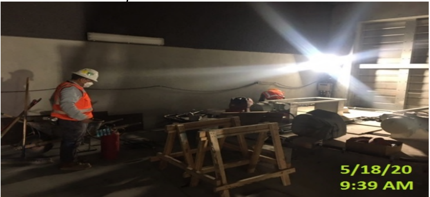
EXPO STATION – Patching and surfacing walls in C-125 Emergency Fan Room North at the concourse level.
