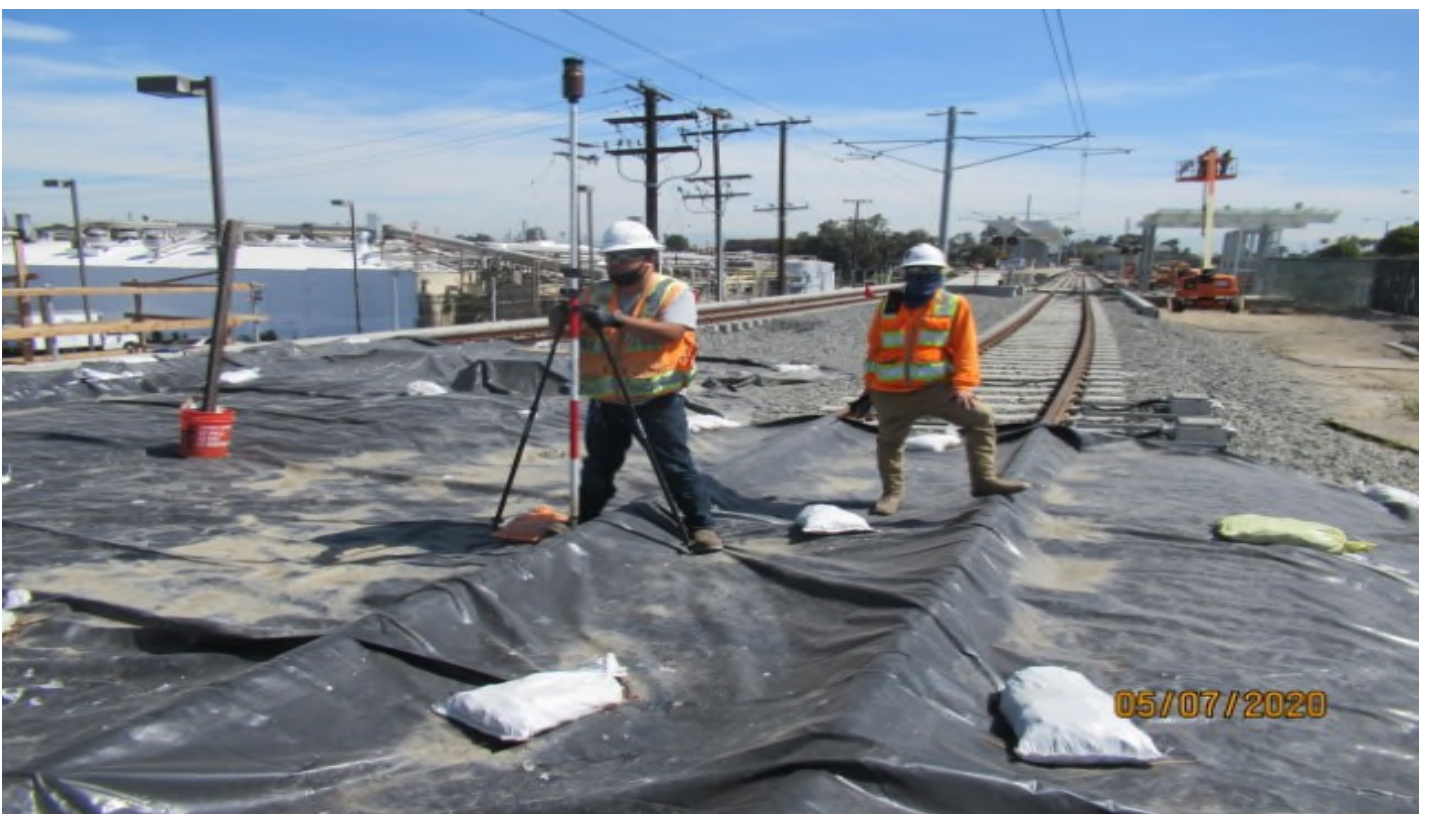
Florence/Brea - Stantec/Metro Surveyors measuring TOR elevations on NB #4 track on La Brea OP STA 206+20
