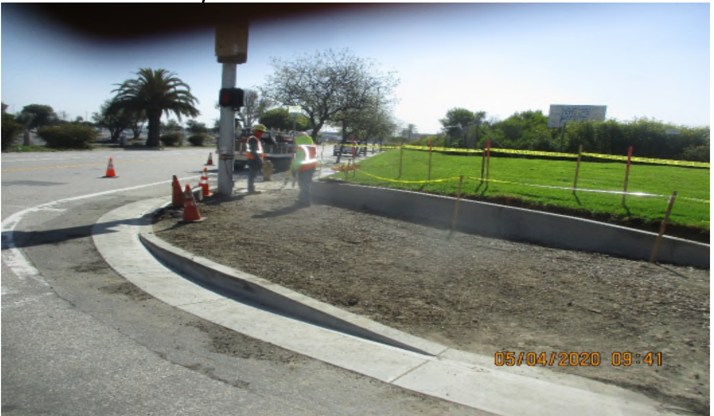
111th Street – WSCC Cut SWK grade at S,E COR of 111Th and Aviation.
