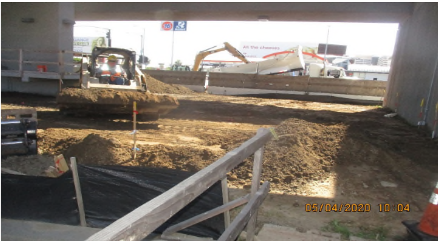
Aviation/Century – WSCC import soil and make grade at S/W COR of Aviation and Century.
