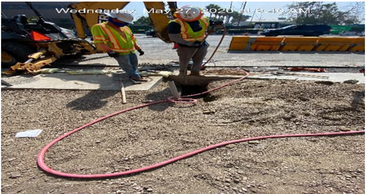
EXPO STATION – Continue excavating for street light foundations and pull boxes on southbound Crenshaw Blvd between Exposition Blvd and Rodeo Blvd.
