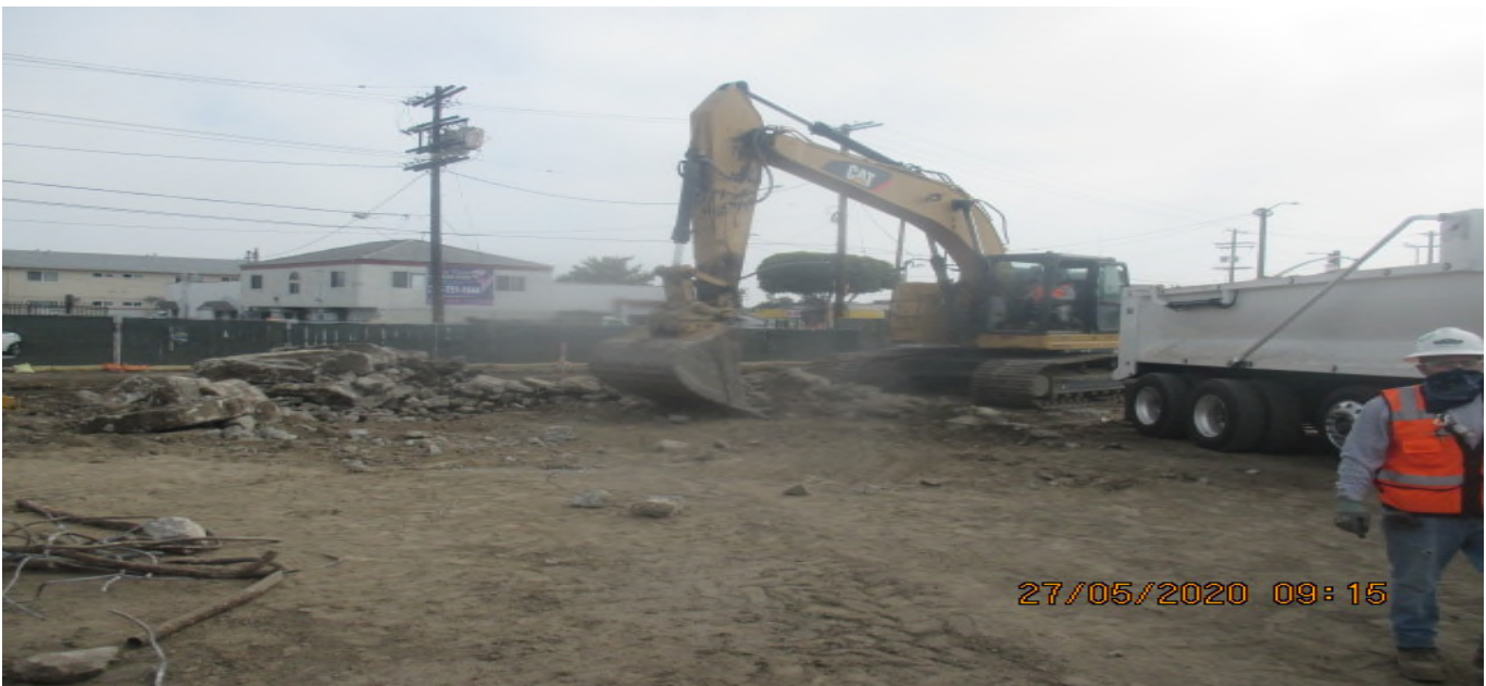
UG3 – Continue excavating the north east section of Victoria Yard for upcoming pavement installation. 5/27/20
