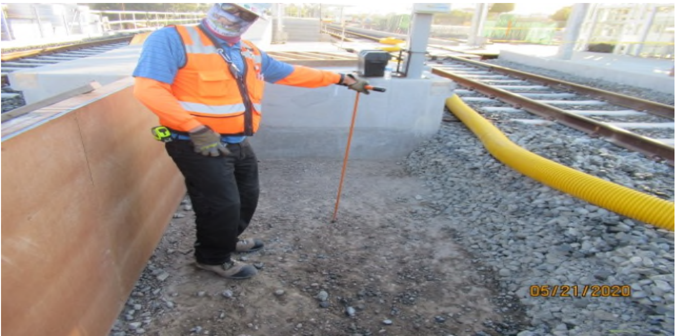
Florence/Brea - WSCC QC inspector verifying sub-ballast compaction on southend of La Brea station platform (outside of track zone of influence)
