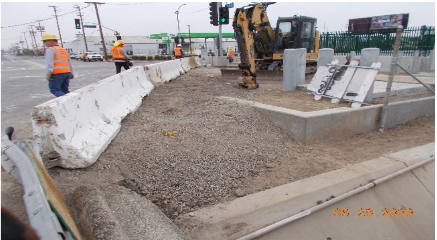
104 th Street - View of excavator that had been compacting dirt on DWP side. 104th.
