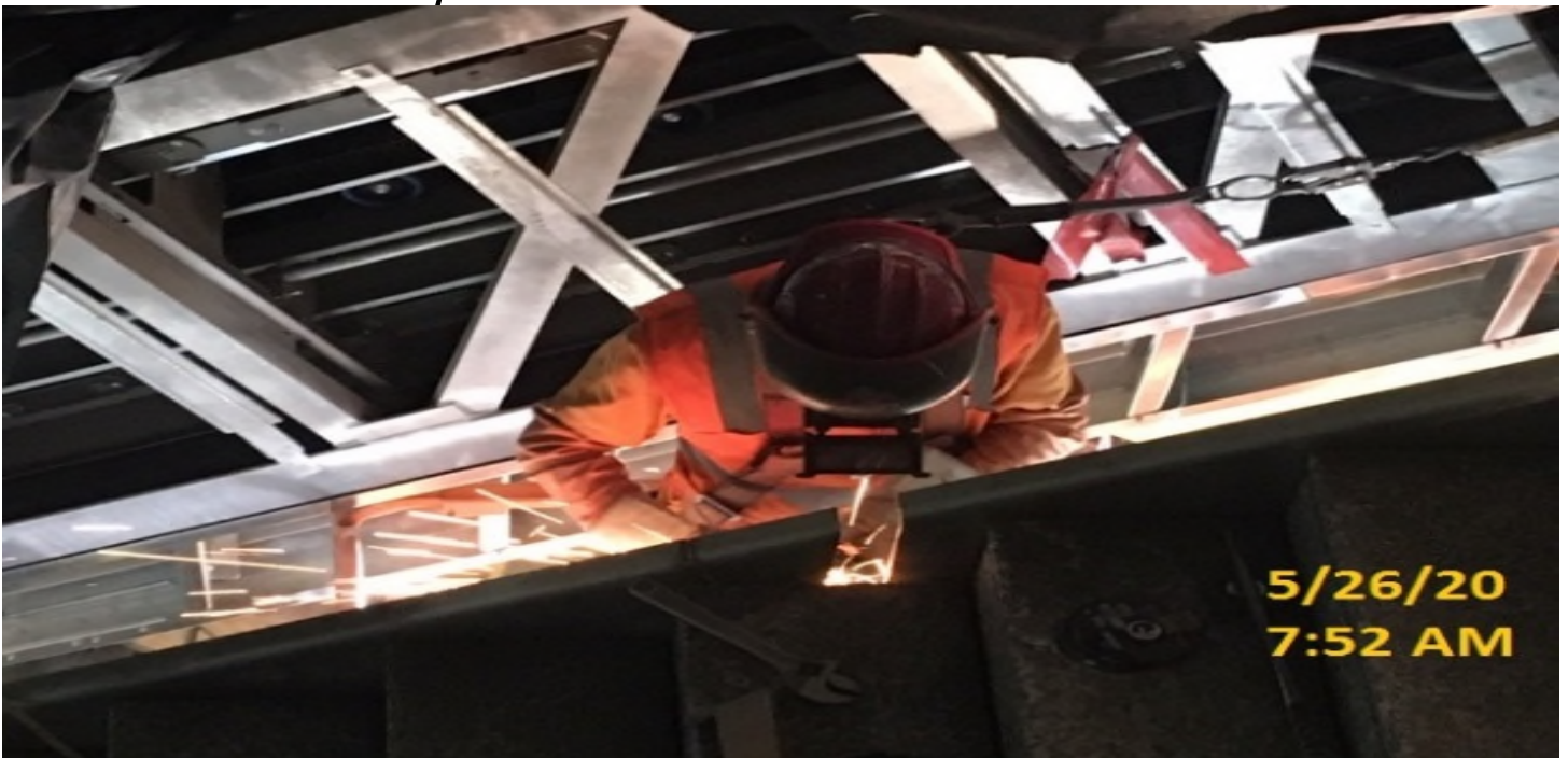
EXPO STATION – Continue cutting/grinding for handrail post installation for staircase #3 from concourse to platform level.
