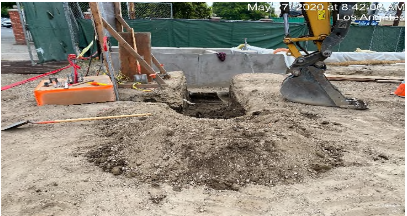
LEIMERT PARK STATION – Continue excavating/trenching for conduit installation throughout the plaza level.
