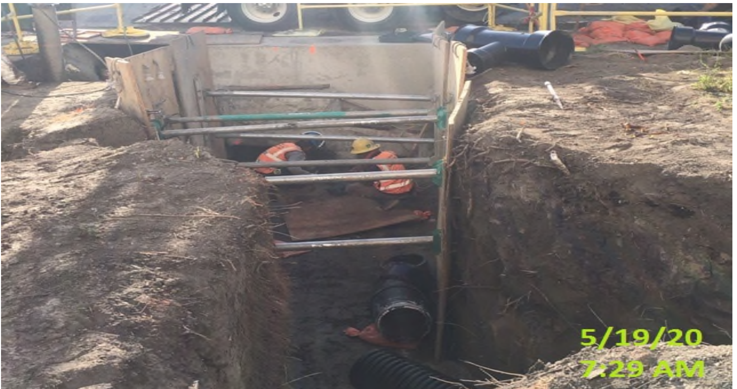
Crenshaw/MLK - MLK – WSCC crew laying 12” HDPE drain line, chipping and potholing for utilities.
