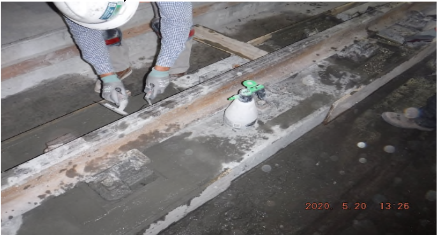
Crenshaw/Expo - STA 447+94 TK#4/NB looking north – left plinth new PCC under DF #3999 and DF #3401 – Exposition Station
