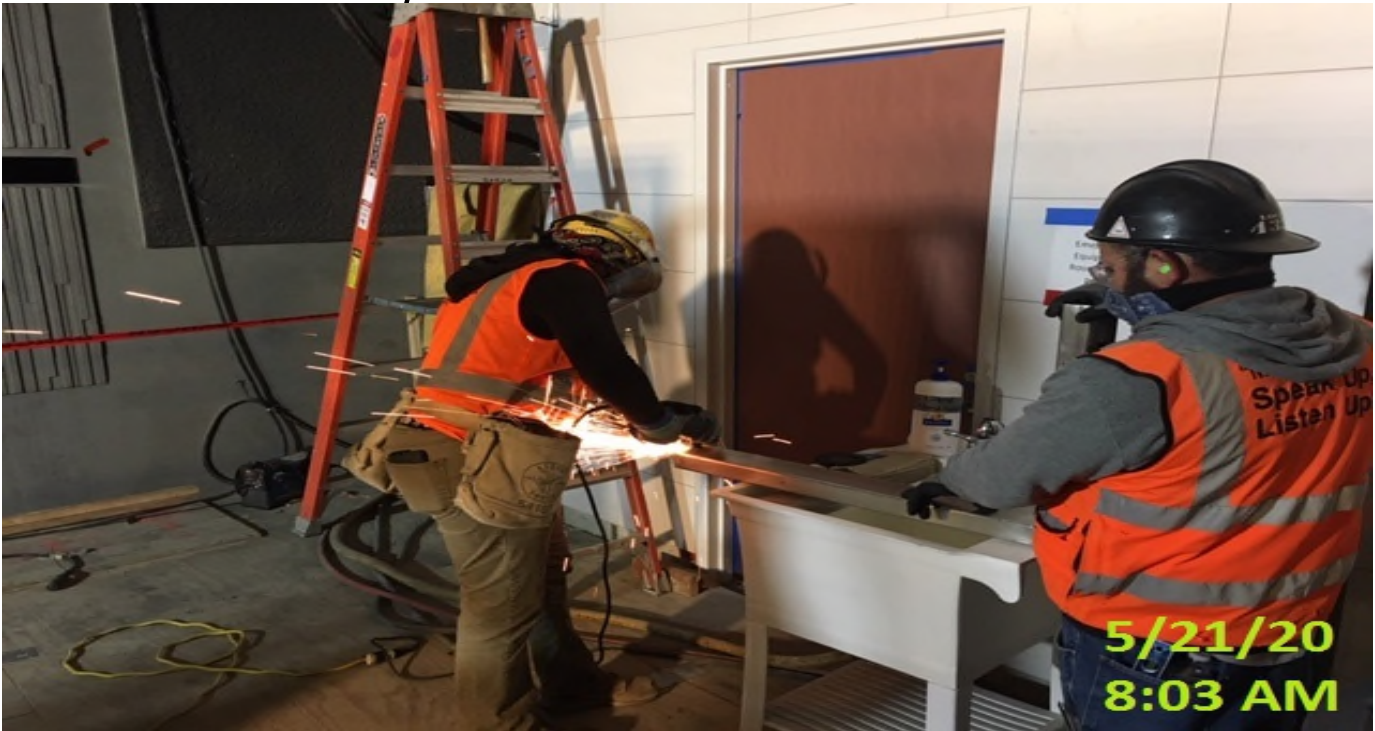
MLK STATION – Grinding header for installation for the north platform end gates on both south and northbound stair landings.
