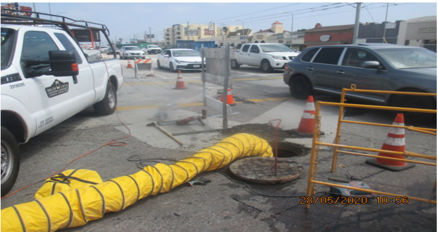
PARK MESA – Sack and patching storm drain line 335 – 2 on southbound Crenshaw Blvd and 57th St. 5/28/20
