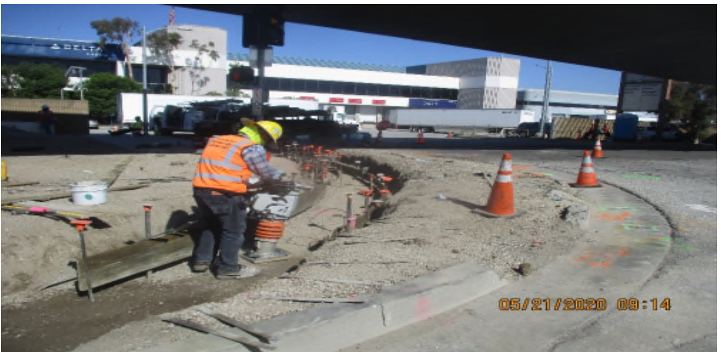
Aviation/Century – Make grade for and place concrete C&G at SW COR of Aviation and 111Th St
