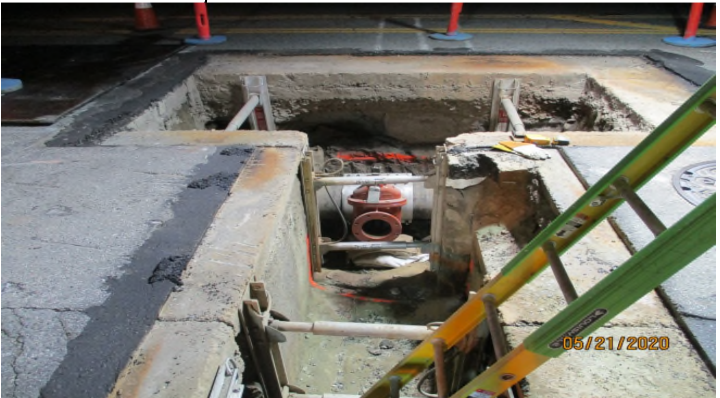
111 th Street – Saddle and valve at the 111th street fire line connection
