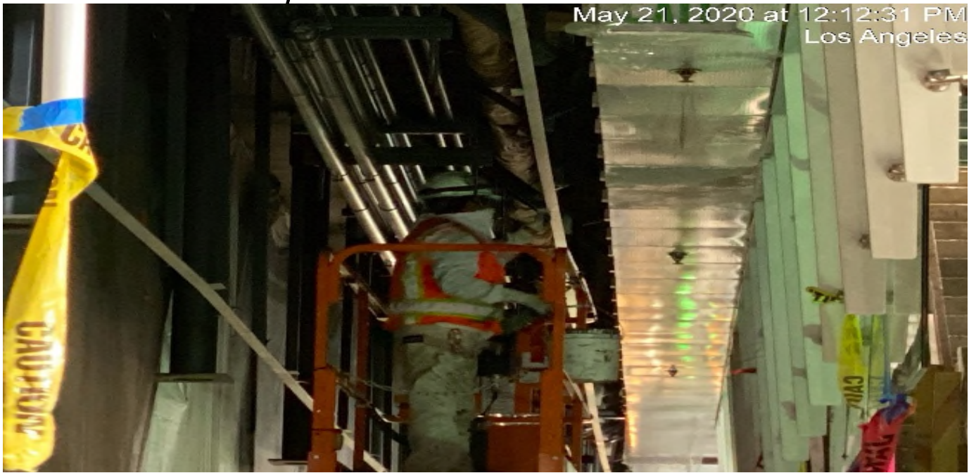
LEIMERT PARK STATION – Continue applying finish paint to the ceiling conduits at the platform level.
