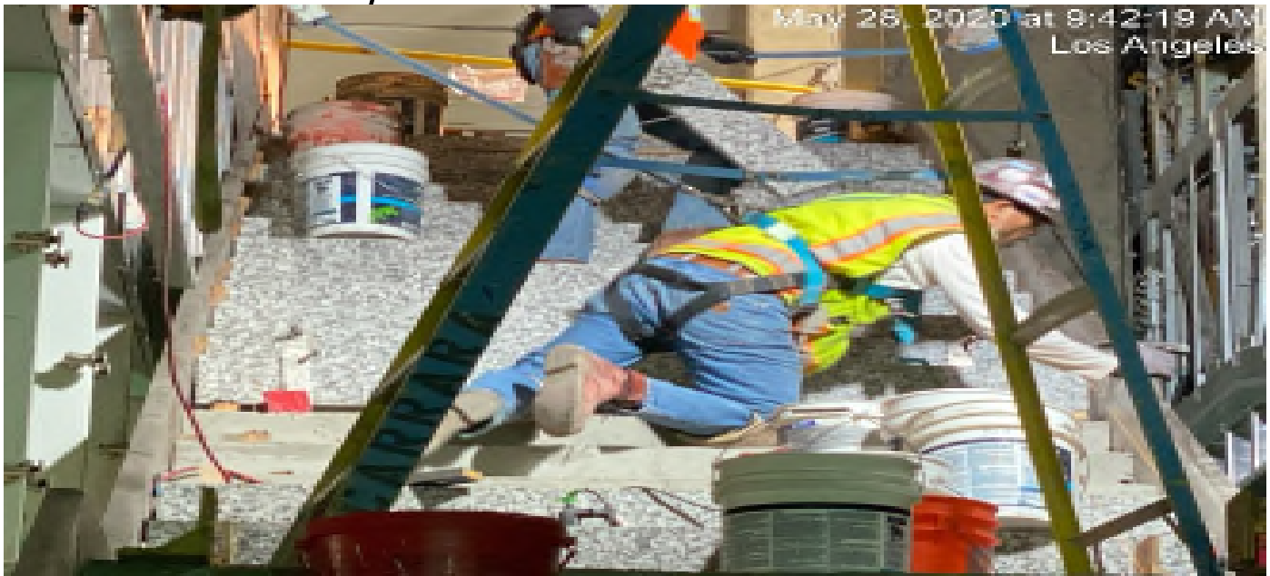
LEIMERT PARK STATION – Continue installing granite tread and riser for staircase #4 from concourse to platform level.
