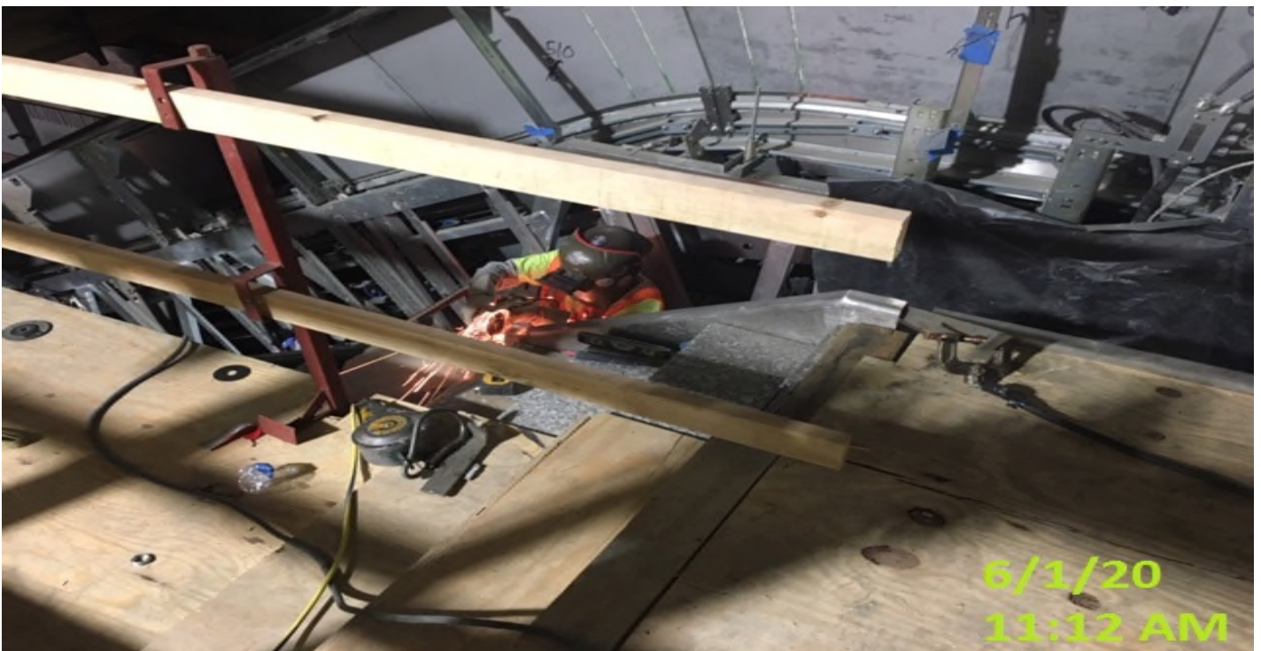
EXPO STATION – Continue cutting/grinding for handrail post installation for staircase #3 from concourse to platform level.
