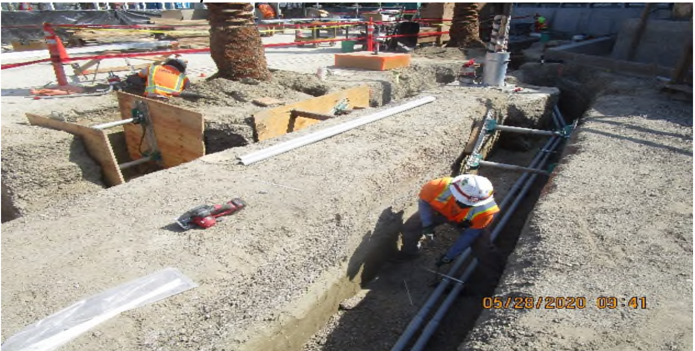
LEIMERT PARK STATION – Began underground conduit installation for landscape lighting for palm trees and canopy at the south side of the plaza level.
