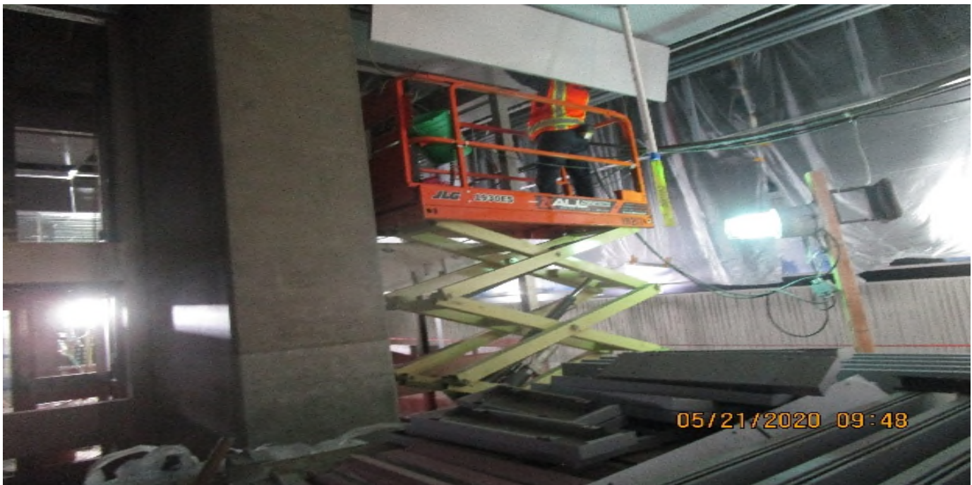
LEIMERT PARK STATION – Resume ceiling light fixture installation at the platform level.
