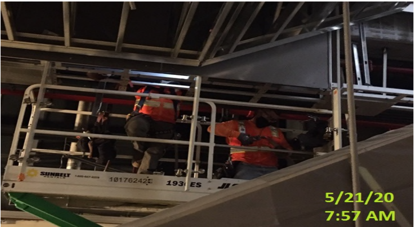
MLK STATION – Continue excavating for new 12” HDPE drainage pipe adjacent to the main entrance canopy structure at the plaza level.
