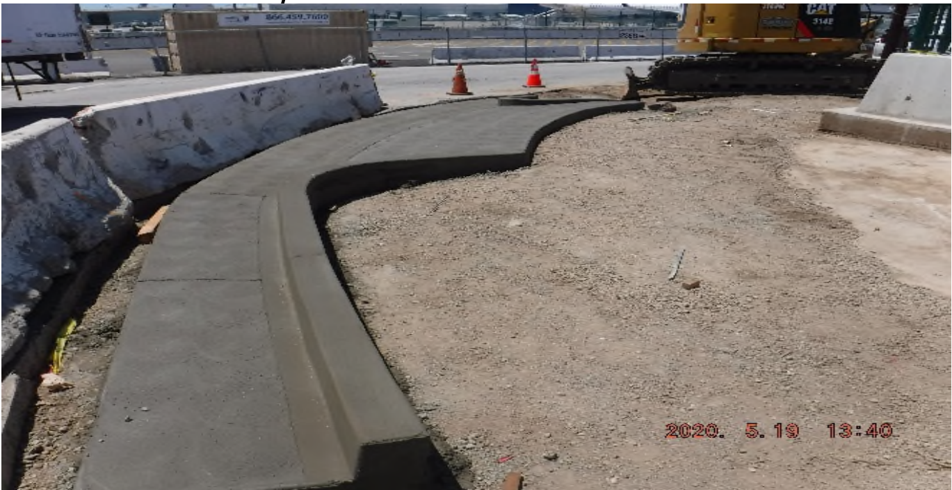
104 th Street - STA 55+25 (TK#4/NB) looking west – new curb return NW corner of 104th St.
