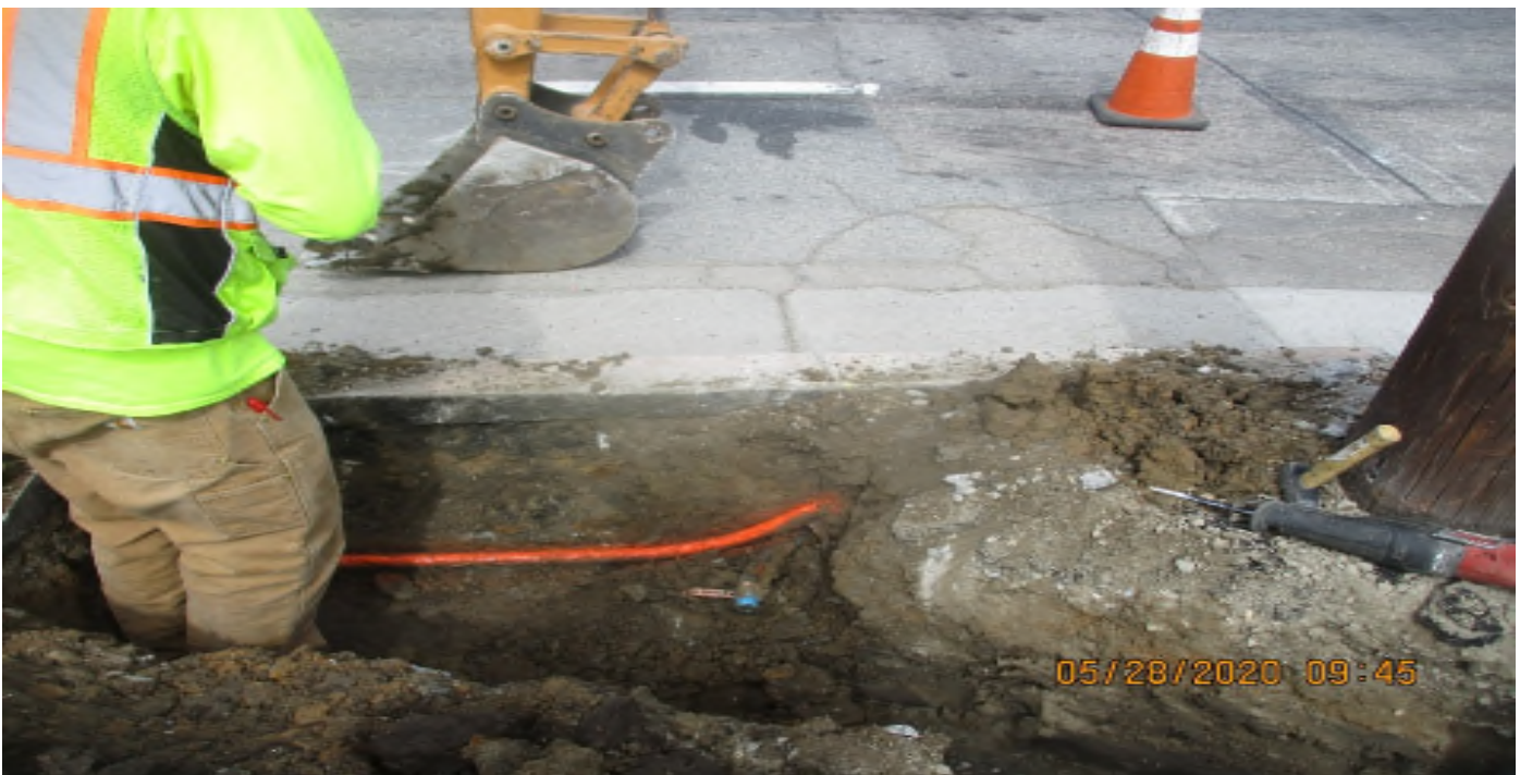
Aviation/Century - DB Electric Found and repaired incomplete conduit at 111th and Aviation.
