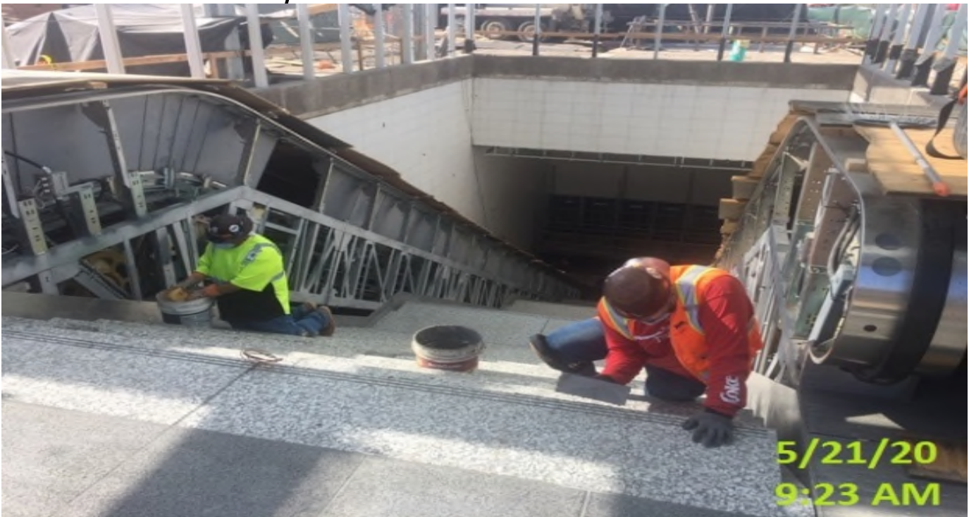
EXPO STATION – Began grouting the granite riser, treads, and stringer tiles at the main entrance staircase.
