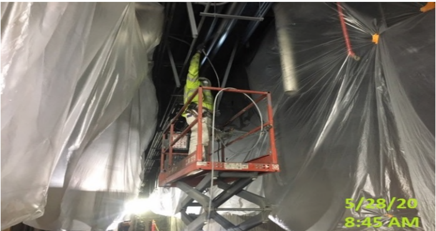
EXPO STATION – Applying finish paint to the ceiling conduit on the platform level.
