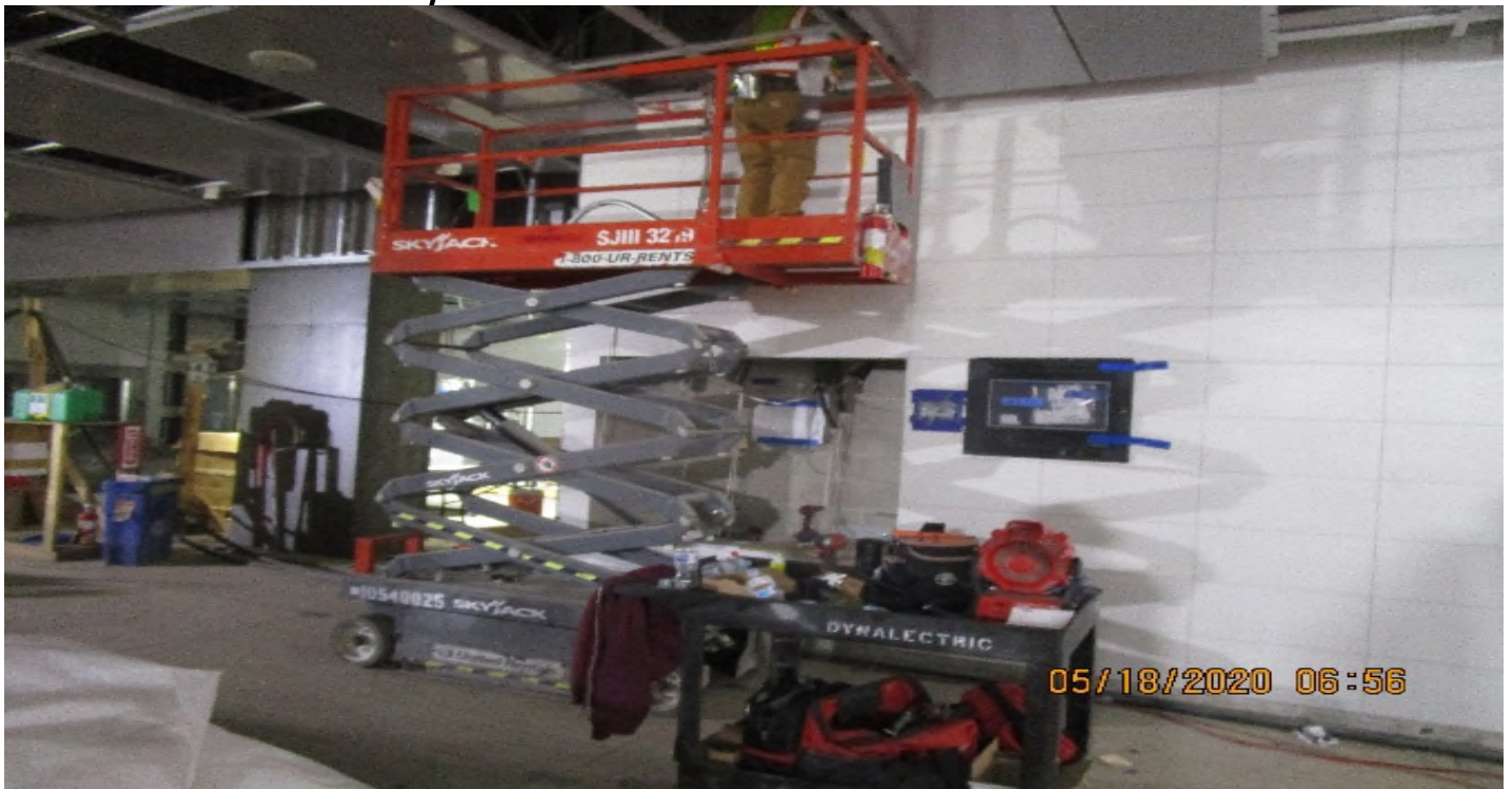
Crenshaw/MLK - MLK, Paid Area C119, continued pipping 1" GRC from stubbed ups at CMU feed to Interactive Fire Fighter Display.
