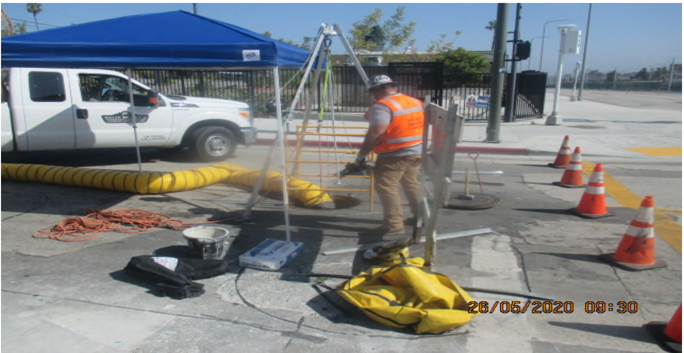
PARK MESA – Sack and patching storm drain line JS-2 on southbound Crenshaw Blvd and 52nd St. 5/26/20
