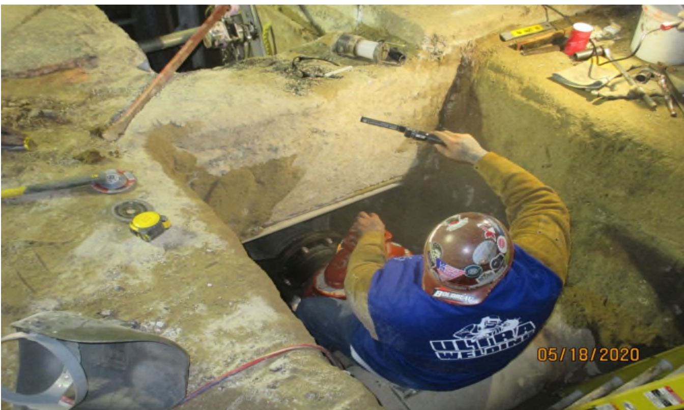
104 th Street - Fabricating the flange to make the fire line connection at 104th street.
