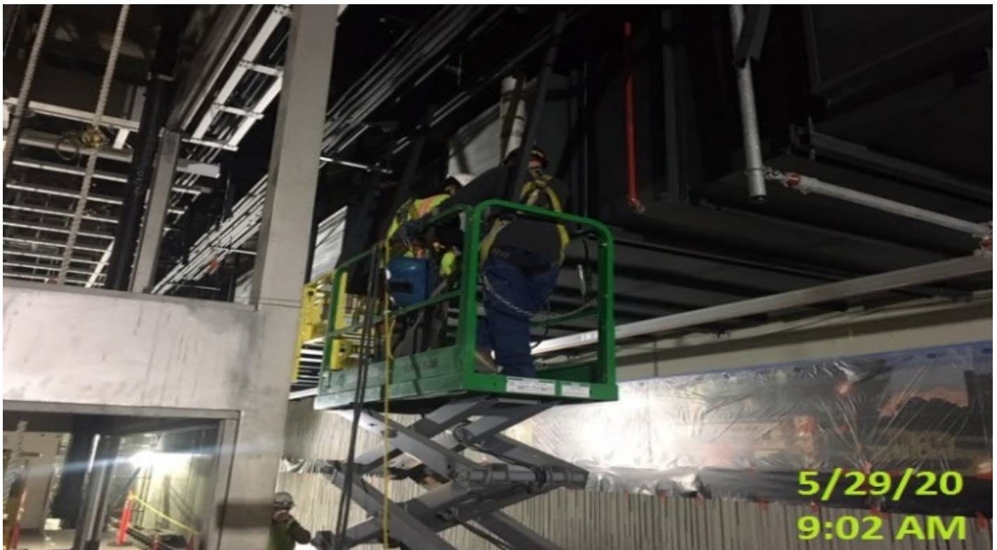
Crenshaw/Expo - EXPO – WSCC ironworker welding upper plates to support poles for edge lighting.
