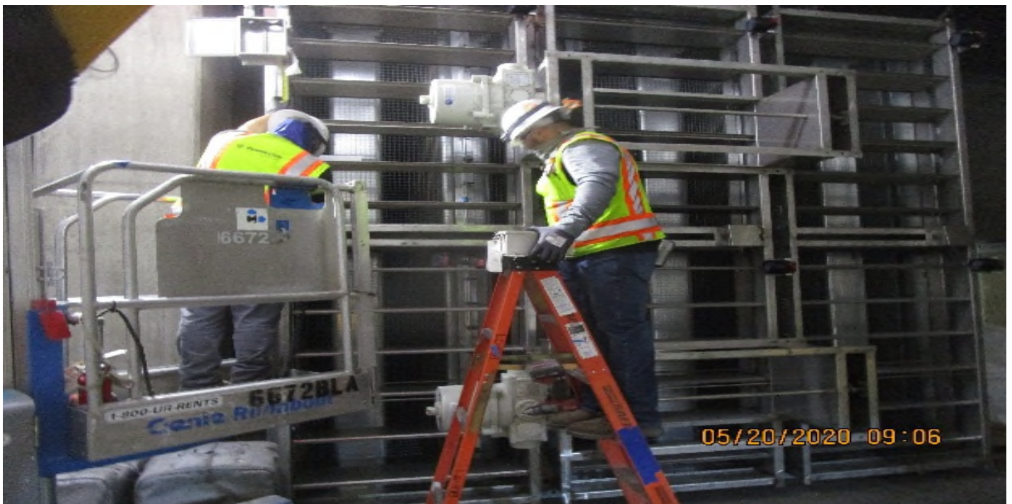
Crenshaw/MLK - MLK, Emergency fan (N) C142, TFD-7-122, Begin rough in Nema-4X JB's, 1" FRP & 3/4" seal tight to limit switches.
