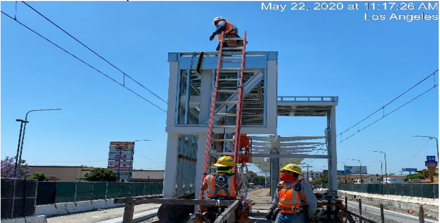
Hyde Park Station – Installing safety cables on top of the north end canopy at the platform level.
