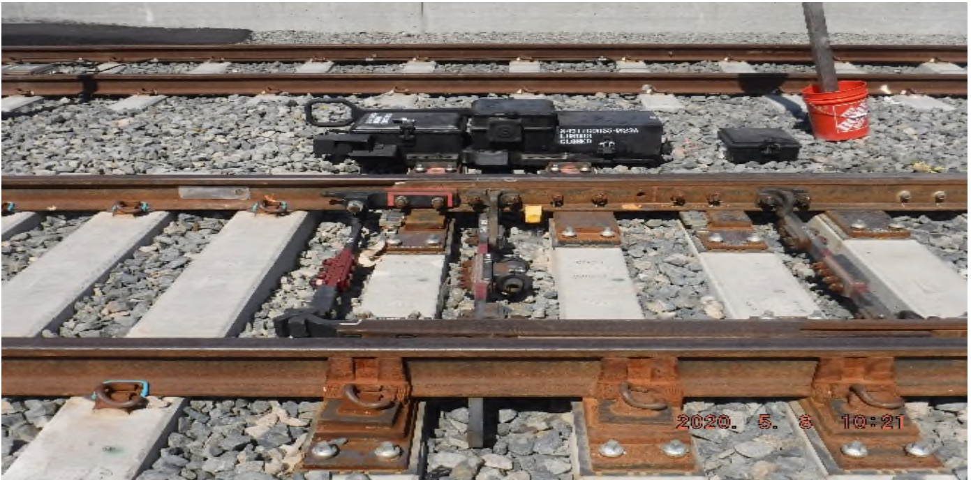
57 th Street - STA 332+54 TK#4,NB looking west – set switch machine on head blocks 10U1LHXO
