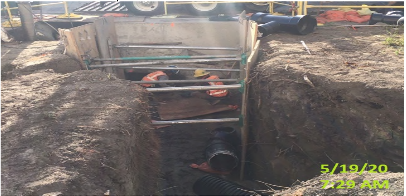
MLK Station - Continue layout of 12” HDPE drainage pipe system connecting to Catch Basin#3 at the northern section of the plaza level.
