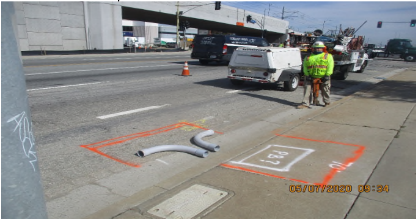
Aviation/Century – DB Electrical Tie in to existing loop circuits at NB Aviation and 104th St.
