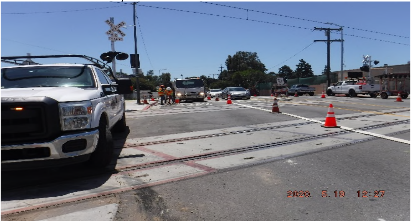
Florence/West – STA 268+00 TK#3/SB looking east – set road / vehicular traffic loop detectors on West Blvd.
