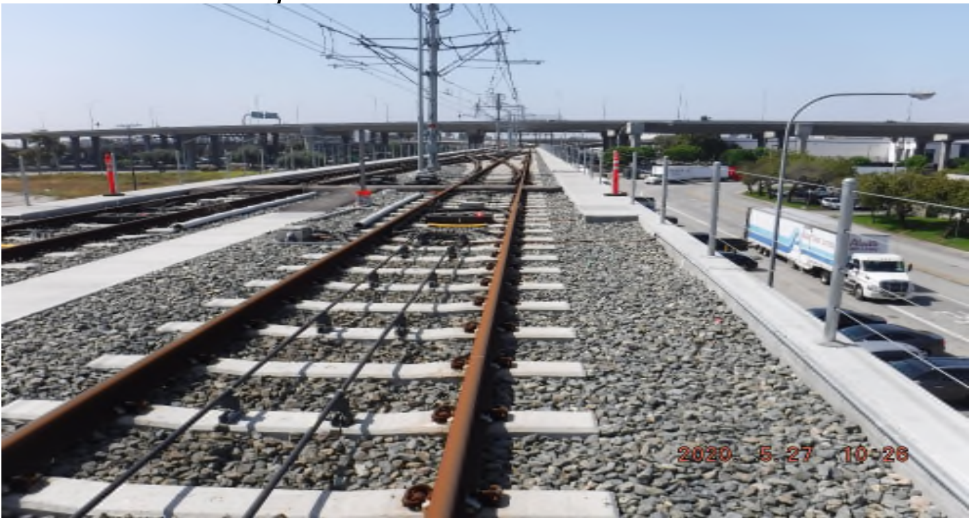
Aviation/Century – 1. STA 21+48 TK#3/SB looking south – rail grind validation in progress (Aviation - DXO area)
