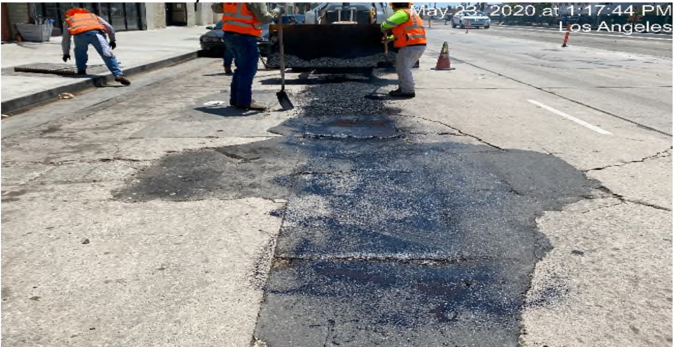
PARK MESA – Asphalt patching various potholes along northbound Crenshaw Blvd between Slauson Ave and 48th St.
