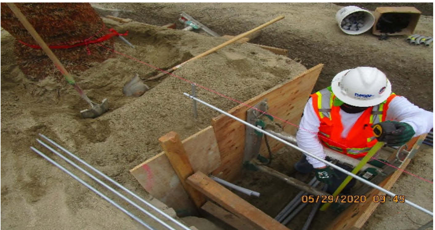
LEIMERT PARK STATION – Continue underground conduit installation for landscape lighting for palm trees and canopy at the south side of the plaza level.
