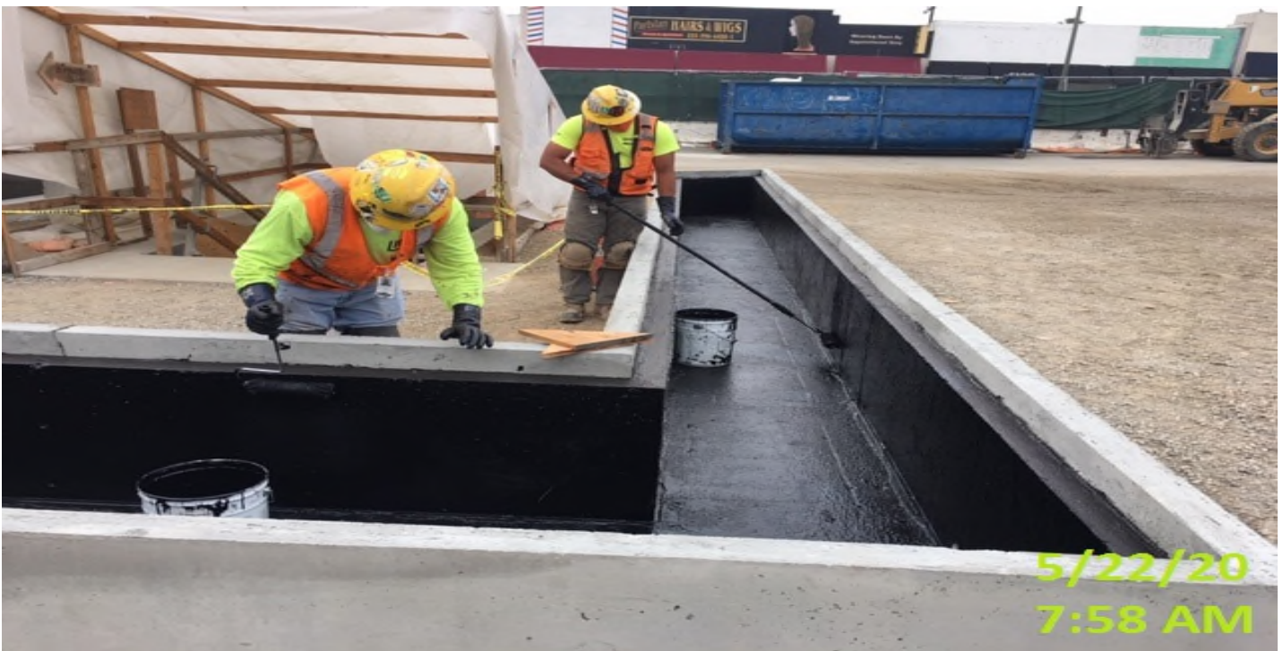
MLK Station - Continue applying waterproofing membrane sealant for the interior of the planter walls at the plaza level.
