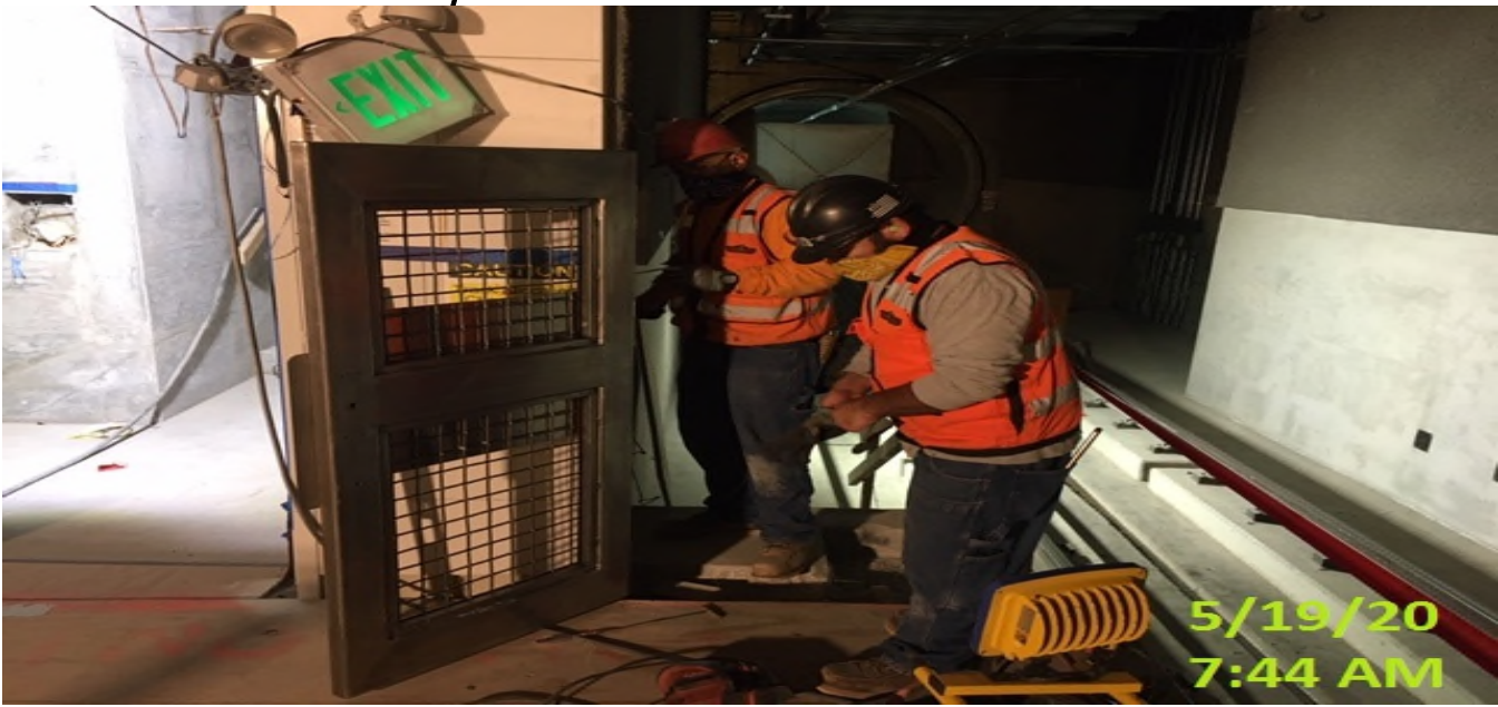
MLK STATION – Excavating for new 12” HDPE drainage pipe adjacent to Elevators 1&2 at the plaza level.
