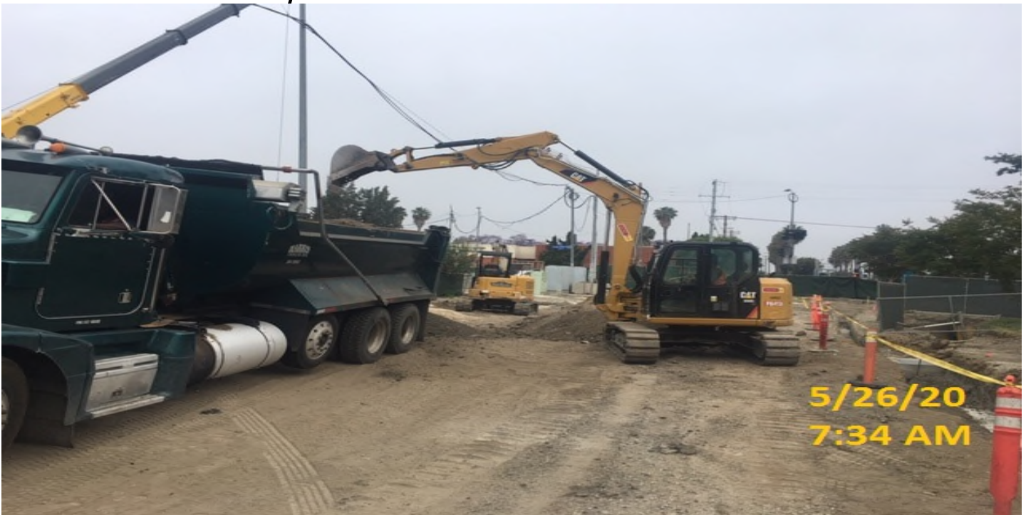
EXPO STATION – Continue excavation/grading for upcoming top soil placement on the north side of the plaza.
