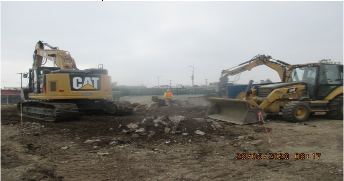
UG3 – Continue excavating the north east section of Victoria Yard for upcoming pavement installation. 5/28/20
