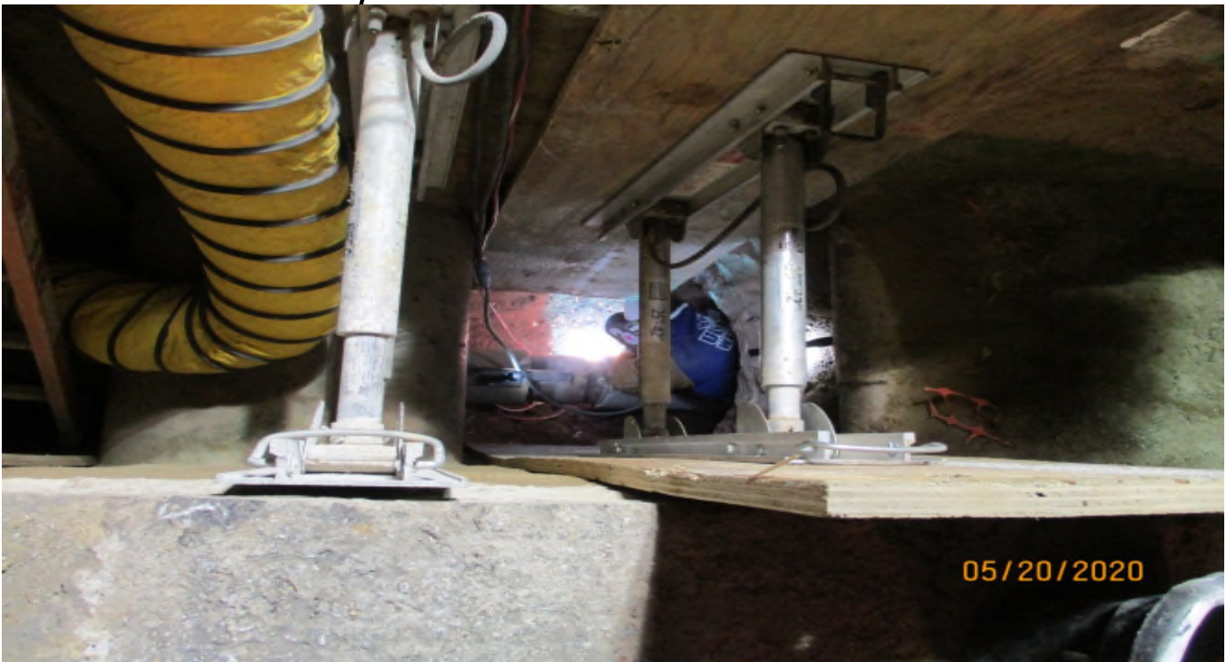
104 th Street - Welding the new section of fire line pipe placed last night at 104th street.
