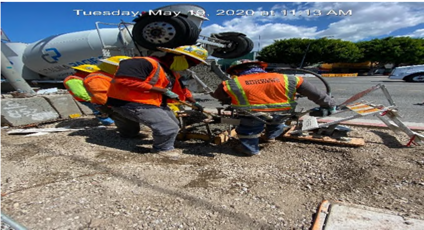
LEIMERT PARK STATION – Build forms and placed concrete for DWP meter boxes on southbound Crenshaw Blvd between Vernon Ave and 43rd Pl.
