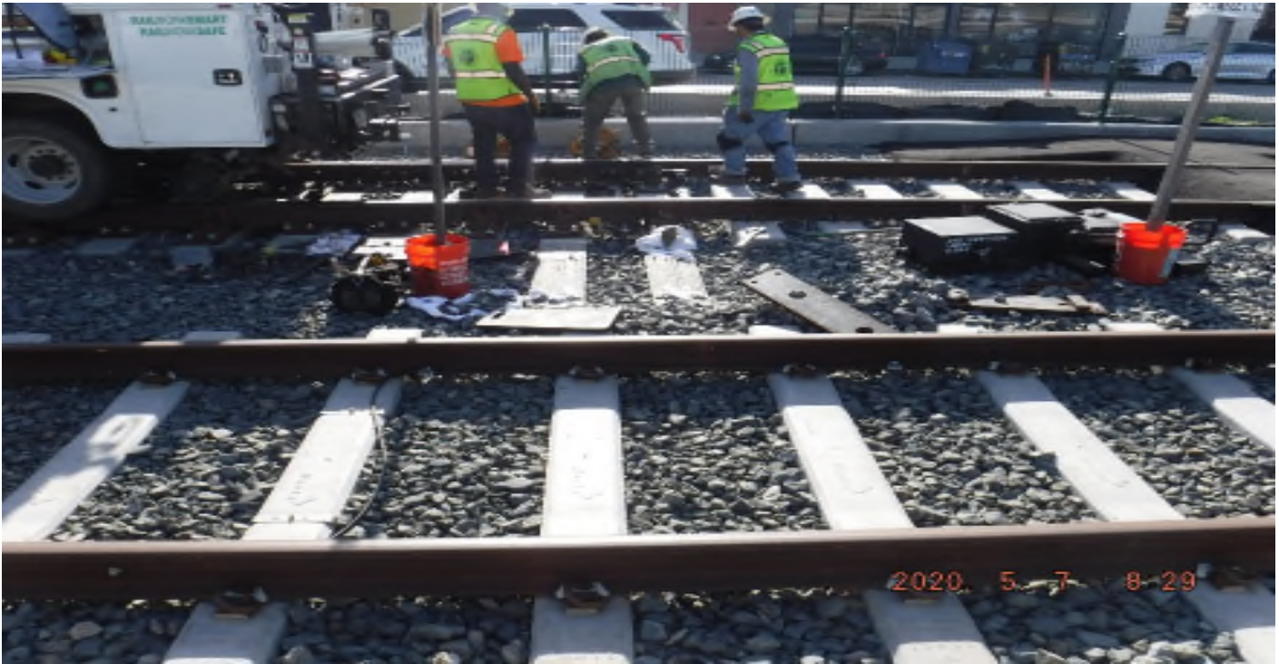
57 th Street - STA 332+54 TK#4/NB looking east – set switch machine on head blocks 10U1LXXO
