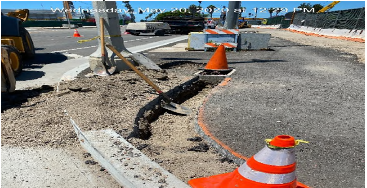
EXPO STATION – Excavating and installing PVC conduit for street light foundations on westbound Rodeo Blvd between Crenshaw Blvd and Bronson Ave.
