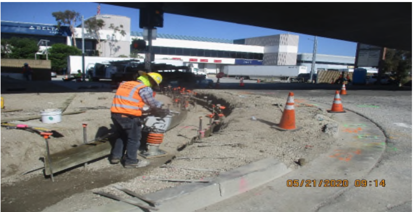
111th Street – Make grade for and place concrete C&G at SW COR of Aviation and 111th St.
