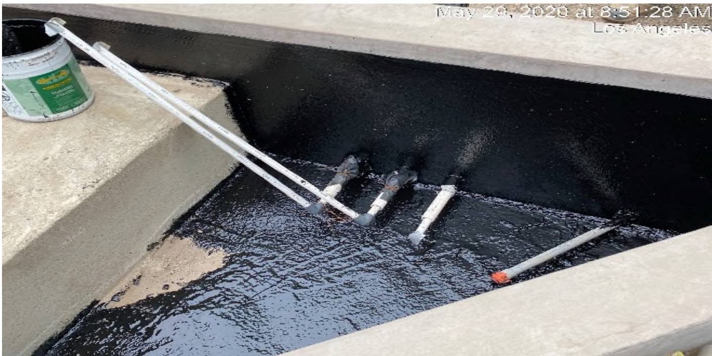
LEIMERT PARK STATION – Applying waterproofing membrane sealant for the interior of the planter walls at the plaza level.
