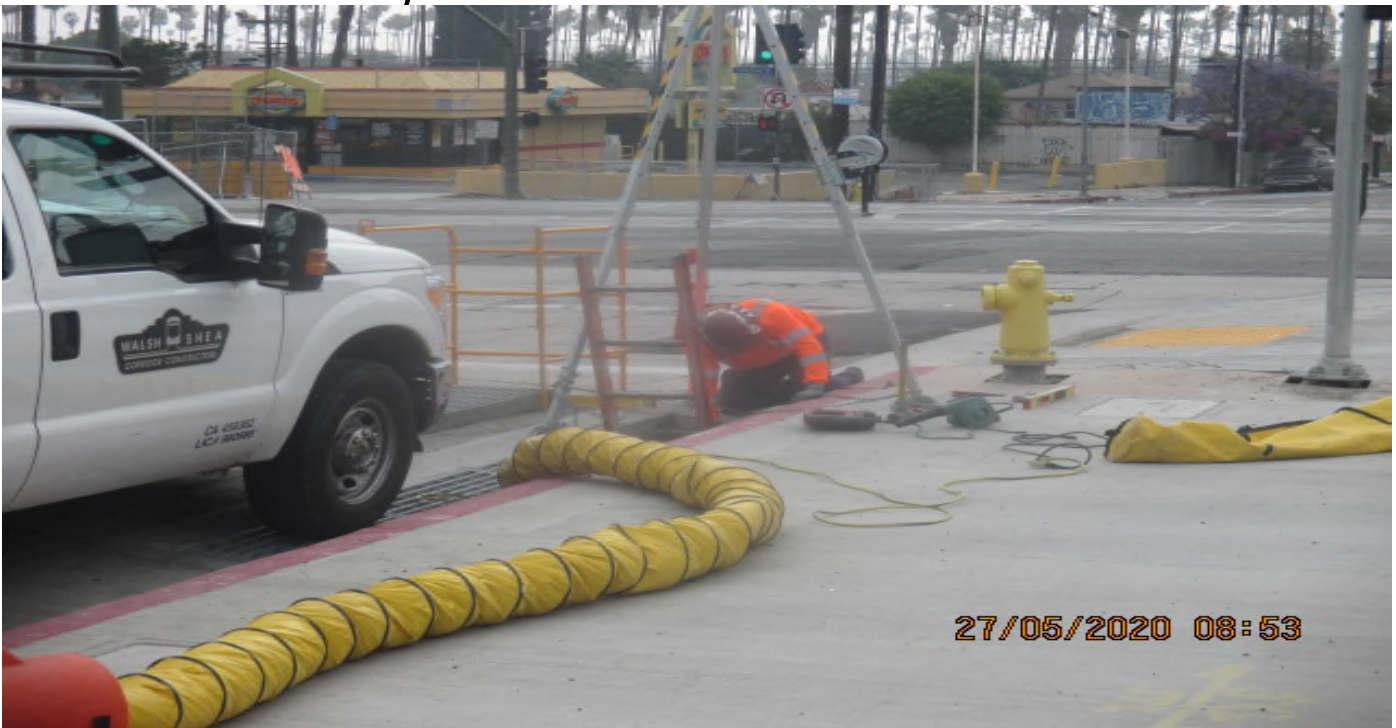
PARK MESA – Drilling and installing ladder rungs inside Catch Basin #27 on the southwest corner of Crenshaw Blvd and 48th St. 5/27/20
