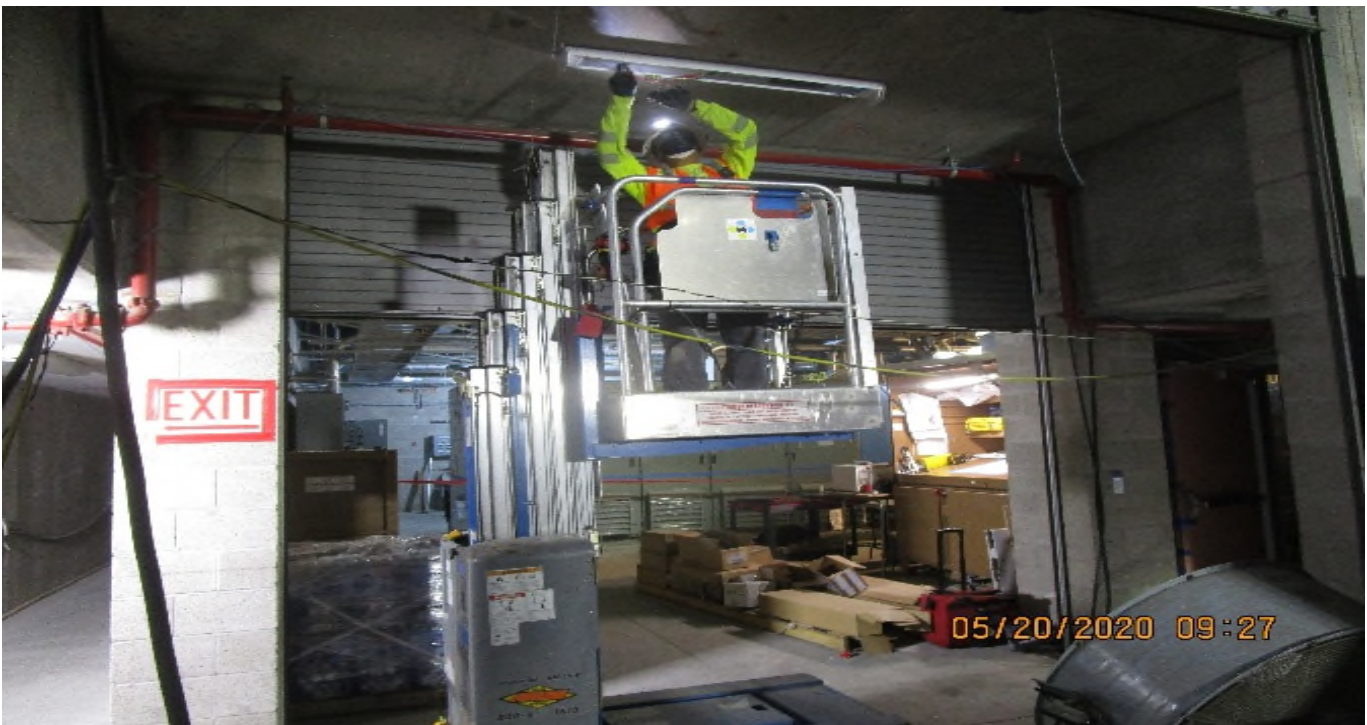
MLK – Began rough-in and terminations for surface mounted light fixtures at the Tunnel Vent Plenum C – 103 of the concourse level.
