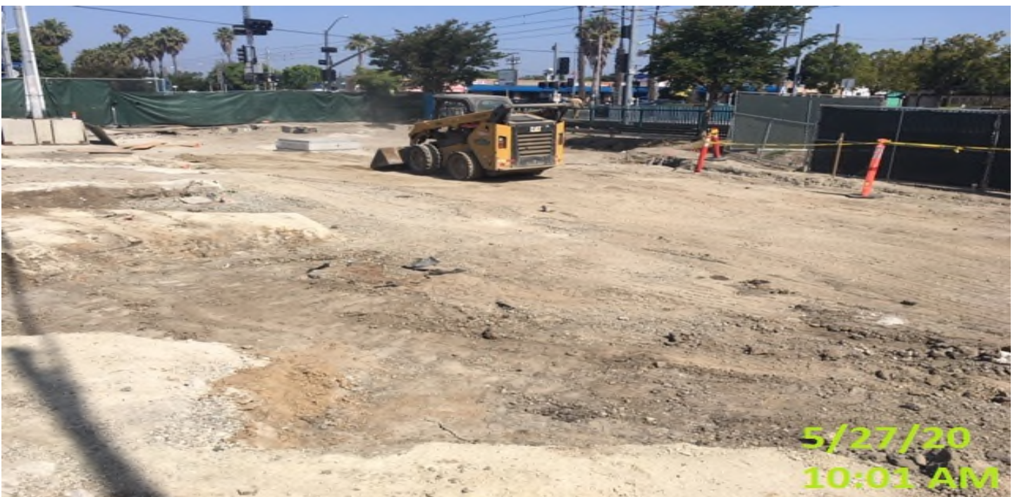
EXPO STATION – Continue excavation/grading for upcoming top soil placement on the north side of the plaza.
