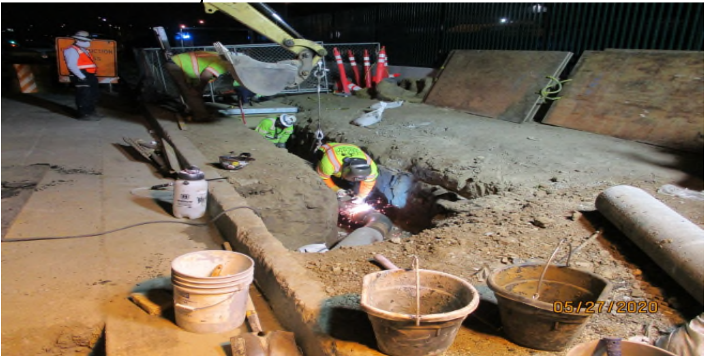
111 th Street – Curb & gutter over-excitation and conduit installation at 111th street. Facing west.
