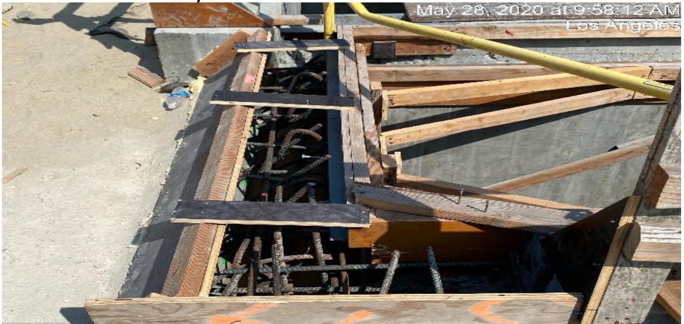
LEIMERT PARK STATION – Continue drilling and doweling for the south emergency exit hatch doors at the plaza level.
