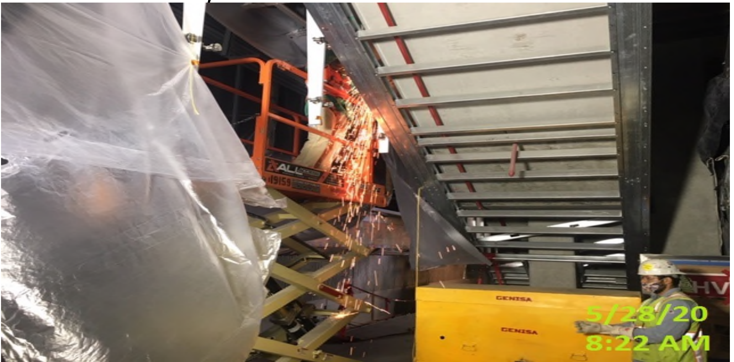
EXPO STATION – Continue cutting/grinding for handrail post installation for staircase #3 from concourse to platform level.
