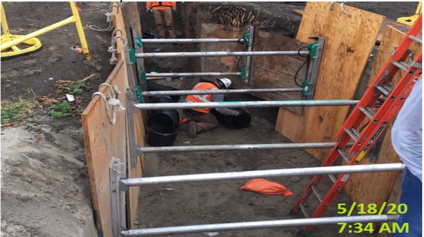
Crenshaw/MLK - MLK – WSCC crew laying 12” HDPE drain line and connecting to catch basin #3
