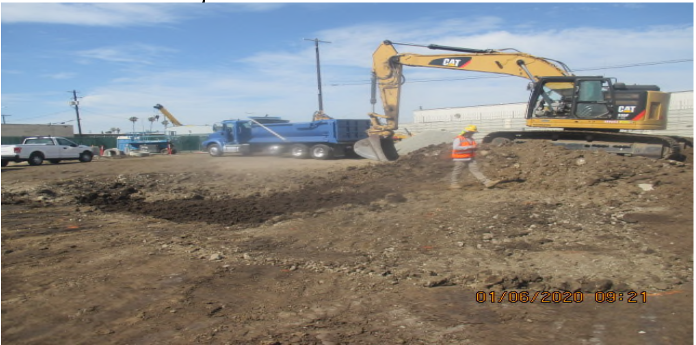
UG3 – Continue excavating the north east section of Victoria Yard for upcoming pavement installation. 6/1/20
