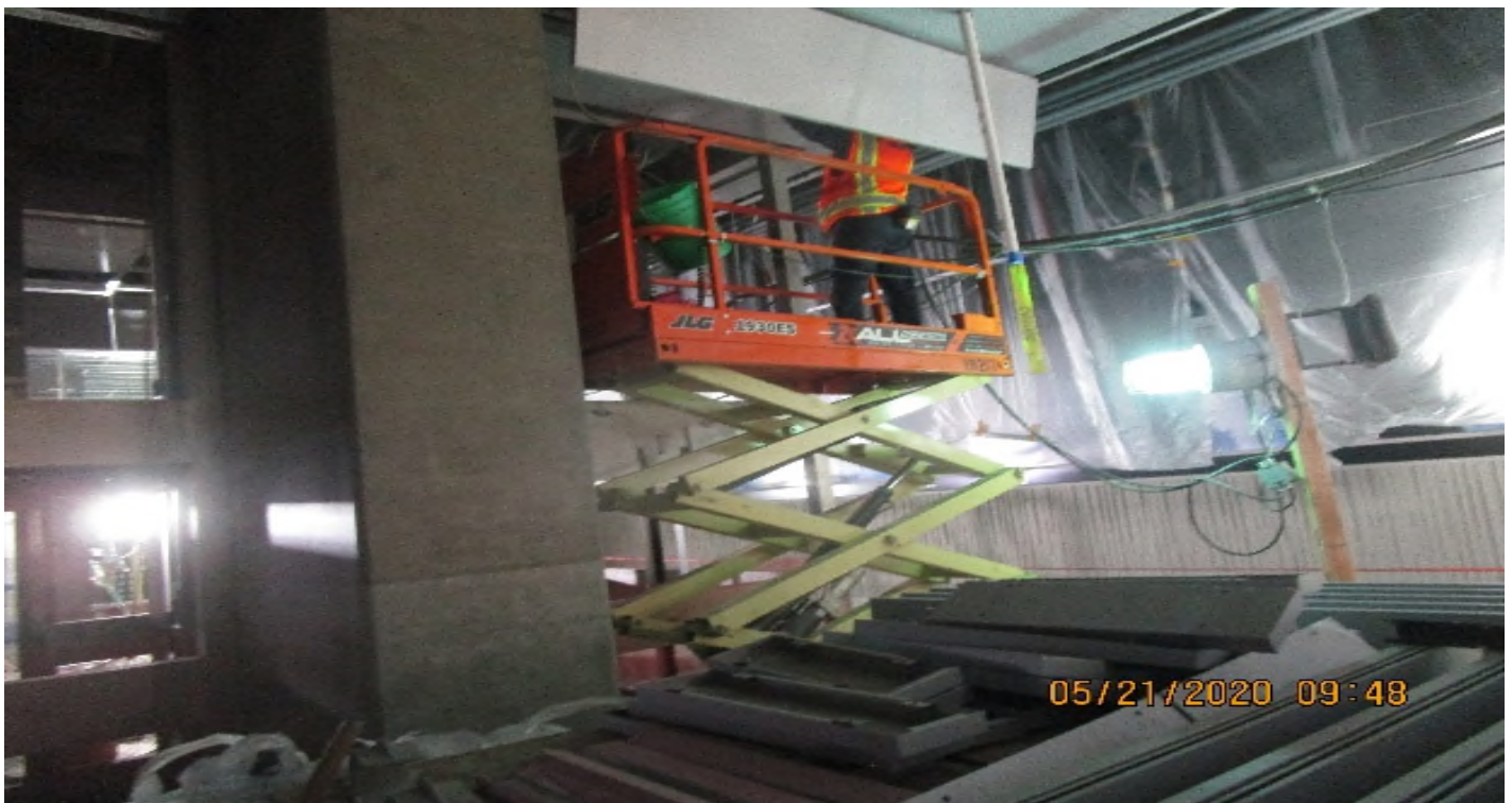
Crenshaw/Vernon - Vernon, GL`s 13-15,A.6-B.4, Overhead resume rough in of Lumium N3-SMF-4-35k-VLO-unu-10D lighting fixtures.
