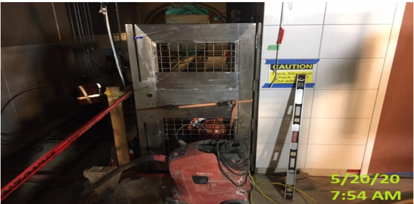
MLK STATION – Continue installing side panels for the north platform end gates on both south and northbound stair landings.
