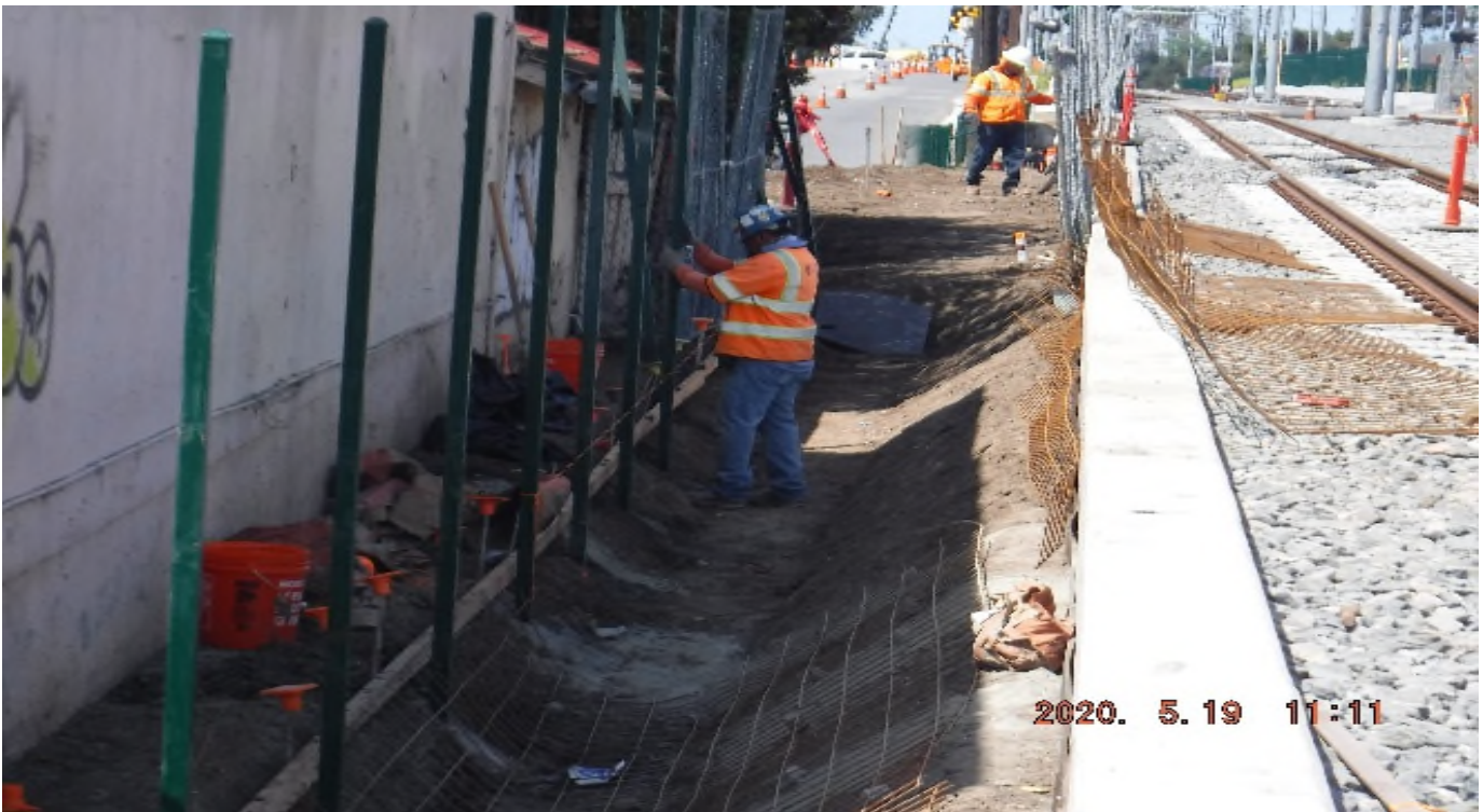
Florence/West – 13. STA 263+00 (TK#4/NB) looking south – fence work along R/W south of West Station.
