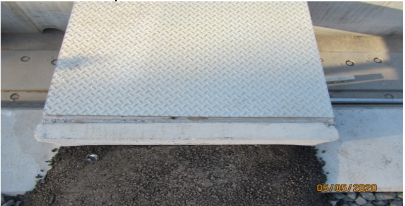
Aviation/Century – Emergency Walkway crossing at edge of DF track on Century/Aviation bridge STA 74+72.
