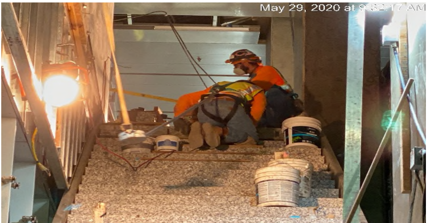
LEIMERT PARK STATION – Continue installing granite tread and riser for staircase #4 from concourse to platform level.
