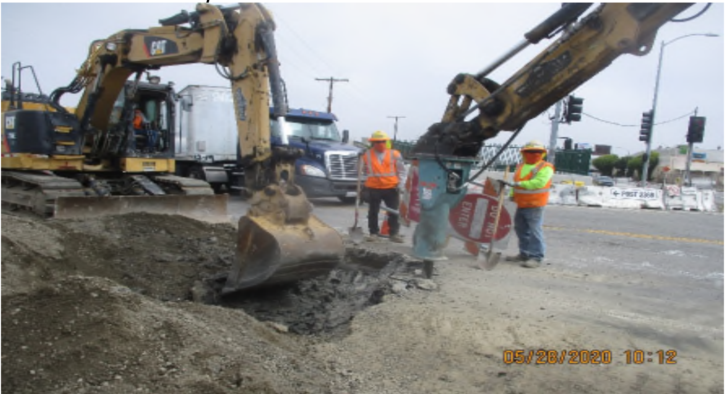
Aviation/Century – WSCC Continued Making removals and C&G Grade at 104th and Aviation.
