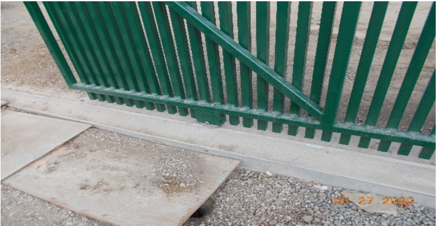
UG3 – Installed track wheels for the sliding gate at the entrance of the Auxiliary Power Bungalow at Victoria Yard.
