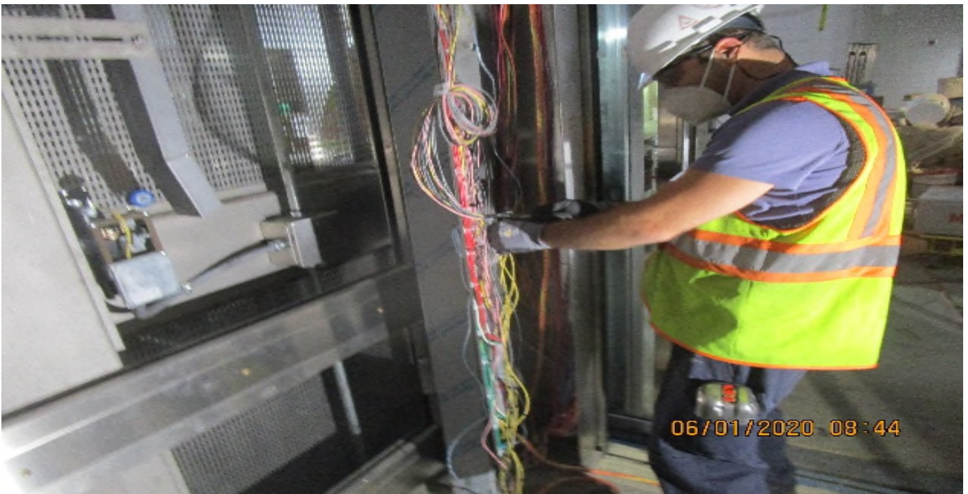
LEIMERT PARK STATION – Continue terminating wires for the cab operating panel for Elevator 2 at the concourse level.
