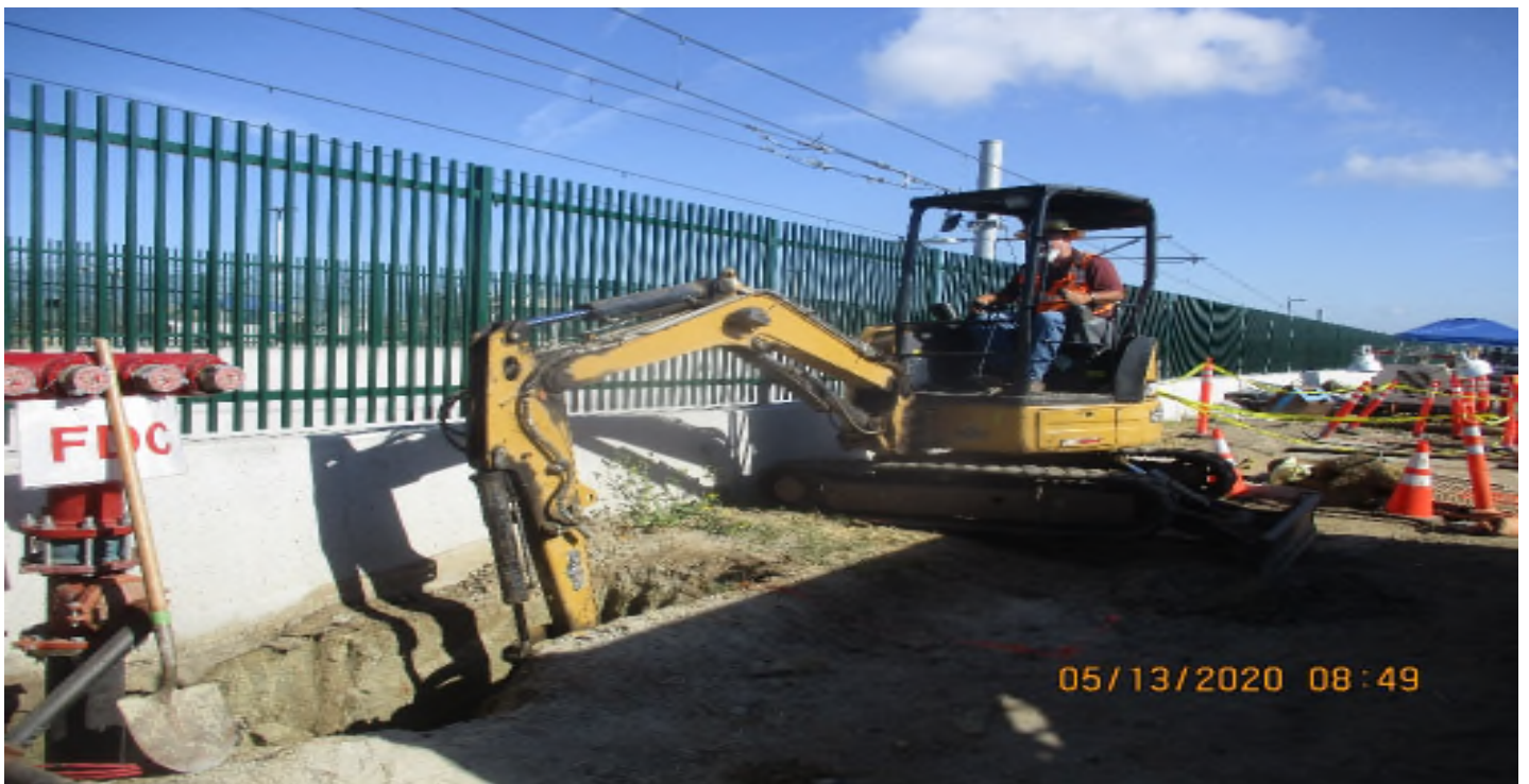
Aviation/Century – WSCC Excavation for Fire line at SB Aviation at end of UG-1.
