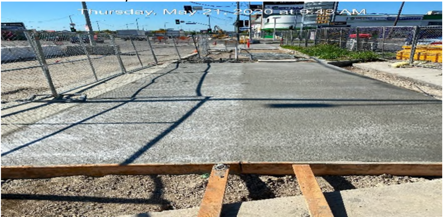
EXPO STATION – Completed driveway on southbound Crenshaw Blvd between Exposition Blvd and Rodeo Blvd.
