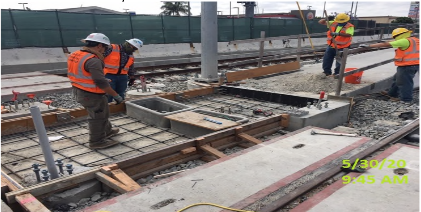
Hyde Park Station – Continue forming and installing rebar for the north end ramp leading to the platform level in preparation for concrete placement.
