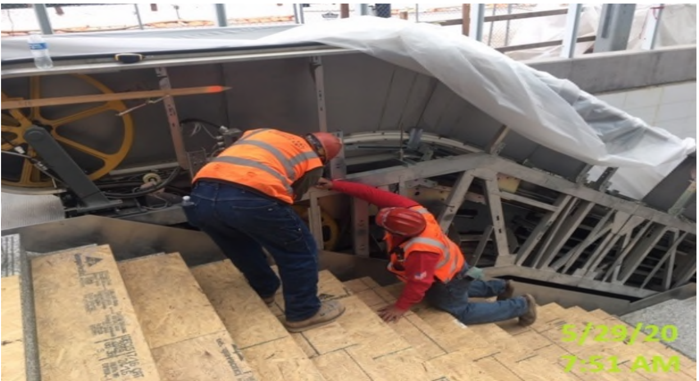
MLK, Measuring layout for upcoming handrail installation for the main entrance staircase at the plaza level.
