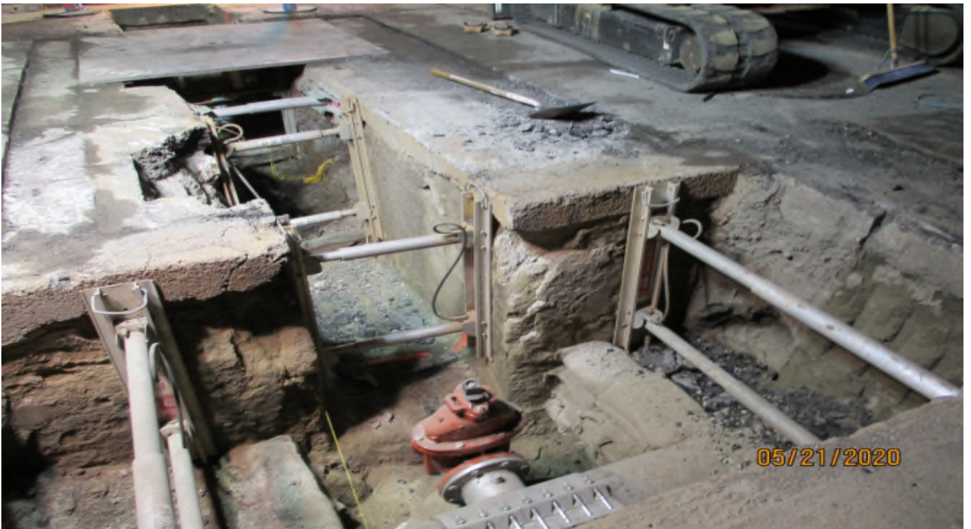
111 th Street – Under mining of the fire line trench at 111th street.
