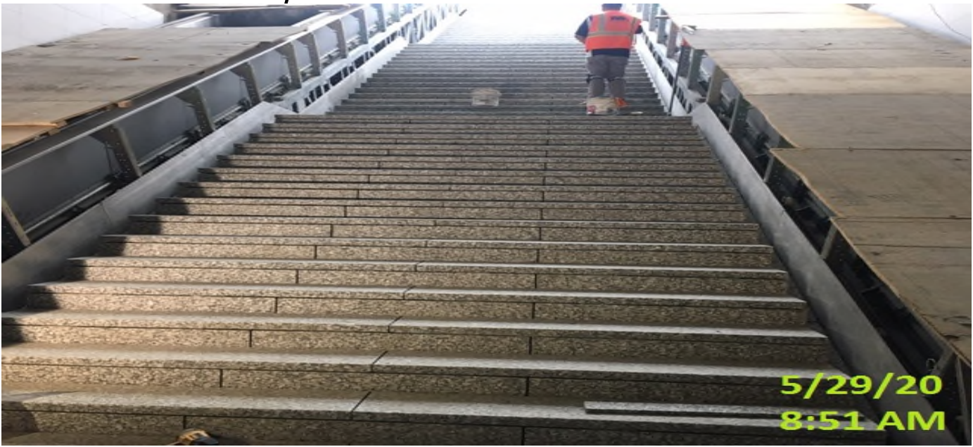
EXPO STATION – Continue grouting the granite risers and treads at the main entrance staircase.
