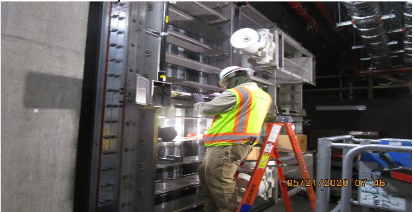
Crenshaw/MLK - MLK, Emergency fan (N) C142, TFD-7-122, Begin rough in Nema-4X JB's, 1" FRP & 3/4" seal tight to limit switches.
