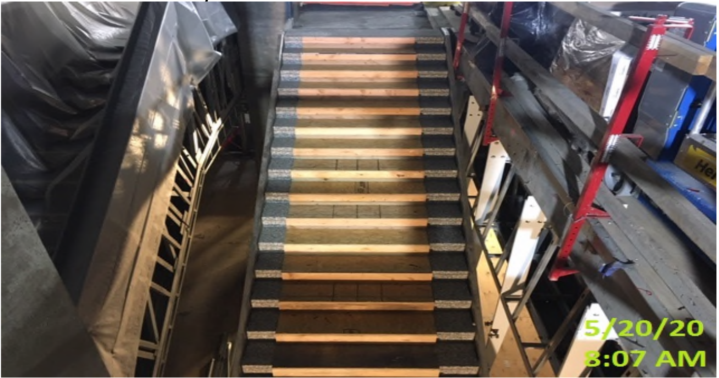
Crenshaw/MLK - MLK – Carrera Marble covering staircase #2 to protect granite risers and treads.
