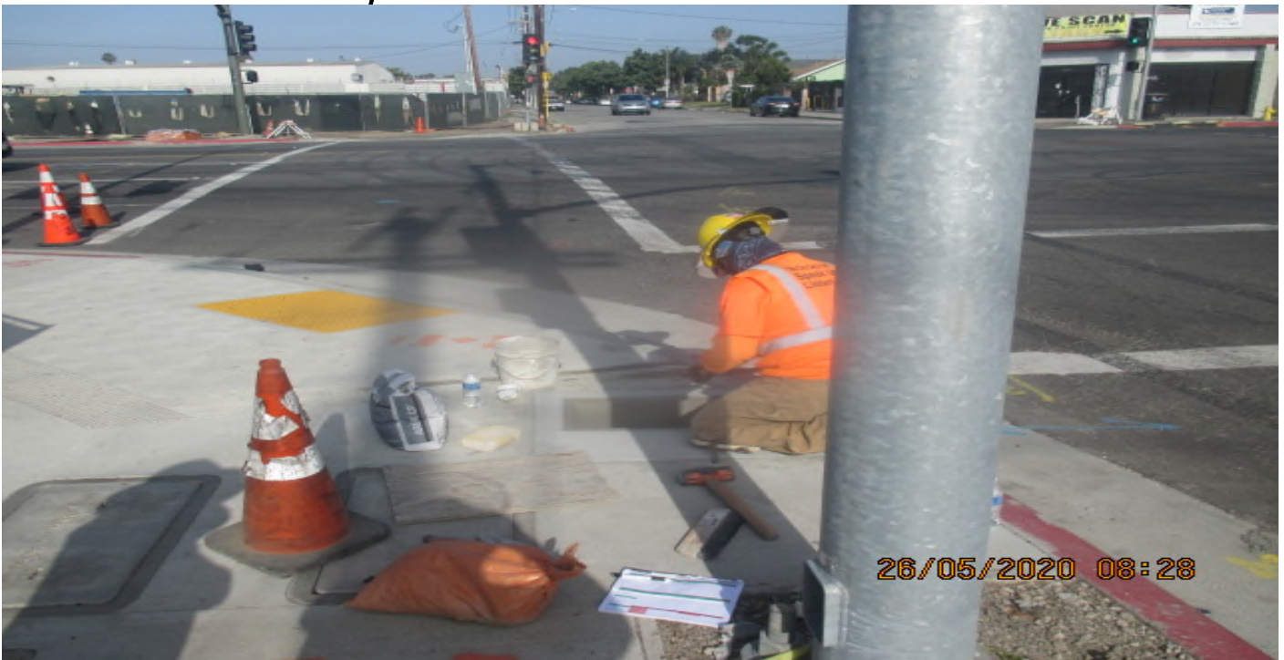
UG3 – Sack and patching DWP water meter box on the southeast corner of 67th St and Crenshaw Blvd. 5/26/20
