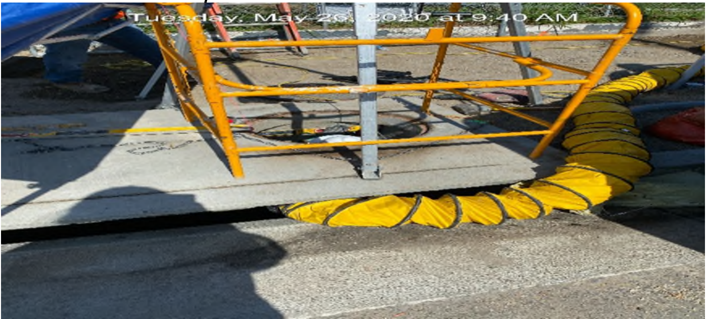
EXPO STATION – Installing steel steps for Catch Basin #16 on southbound Crenshaw Blvd between Exposition Blvd and Rodeo Blvd.
