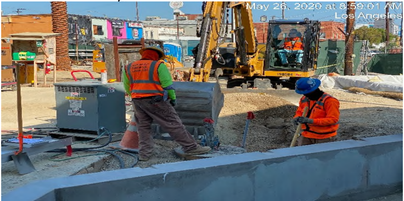
LEIMERT PARK STATION – Continue excavating/trenching for conduit installation throughout the plaza level.
