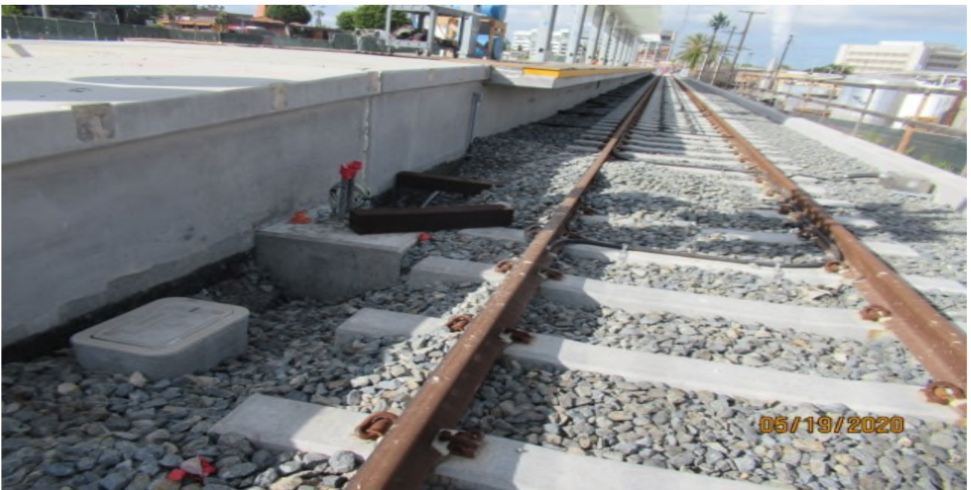
Florence/La Brea – SB #3 track STA 211+07 north side of La Brea station platform, disturbed track ballast, no changes
