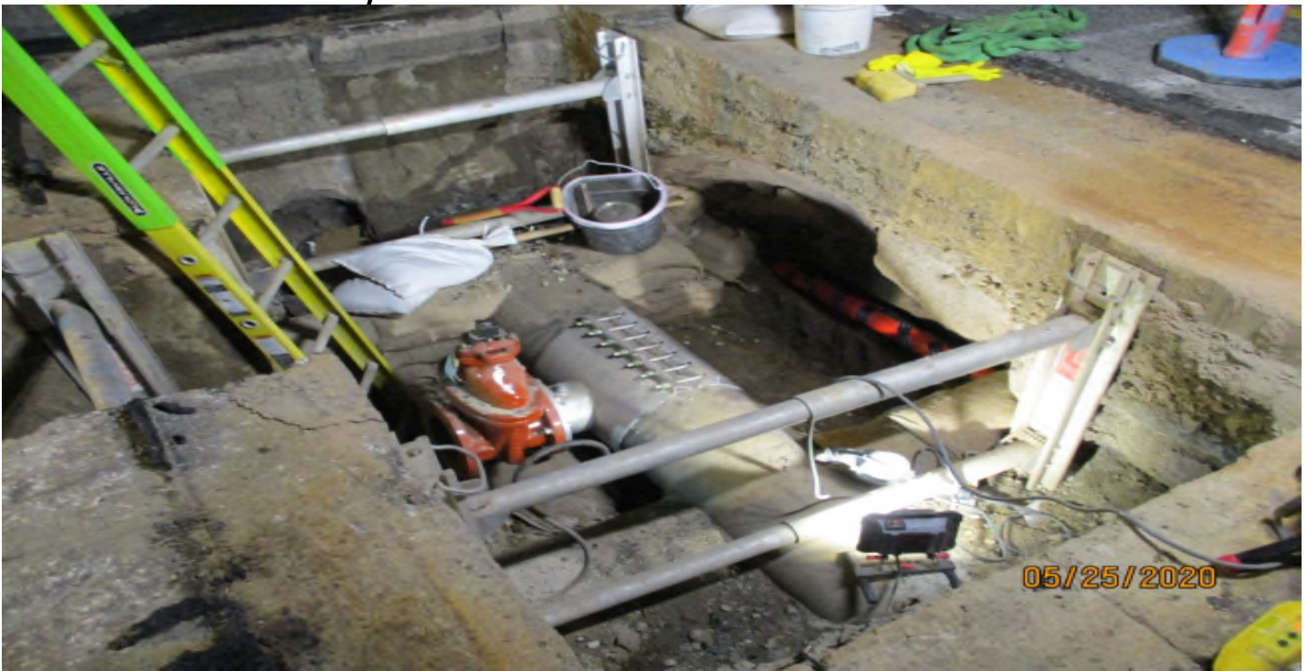
111 th Street – Fire line saddle and valve prior to concrete placed for the thrust block at 111th street.
