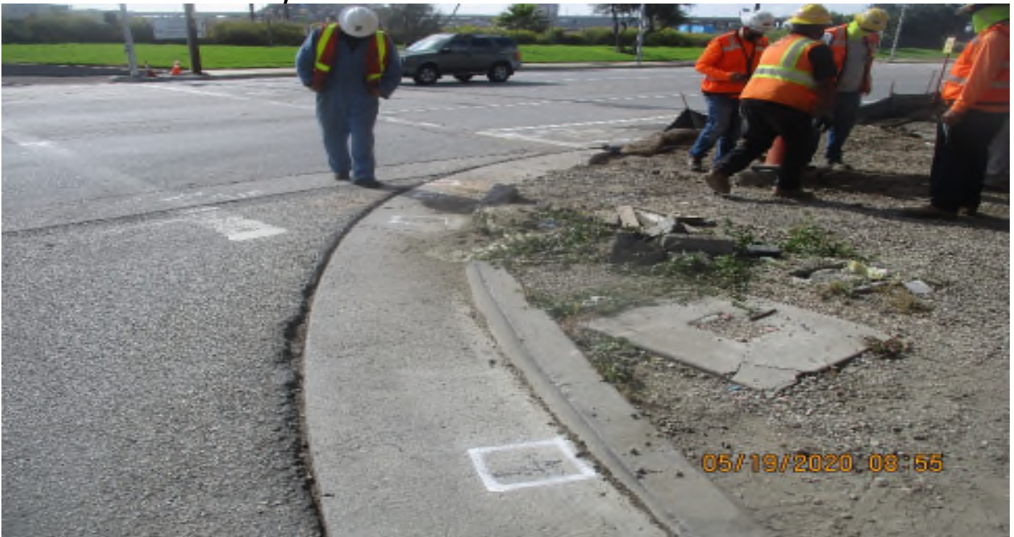
111th Street – WSCC Started removals of old C&G at 111Th and Aviation S/W CORNER
