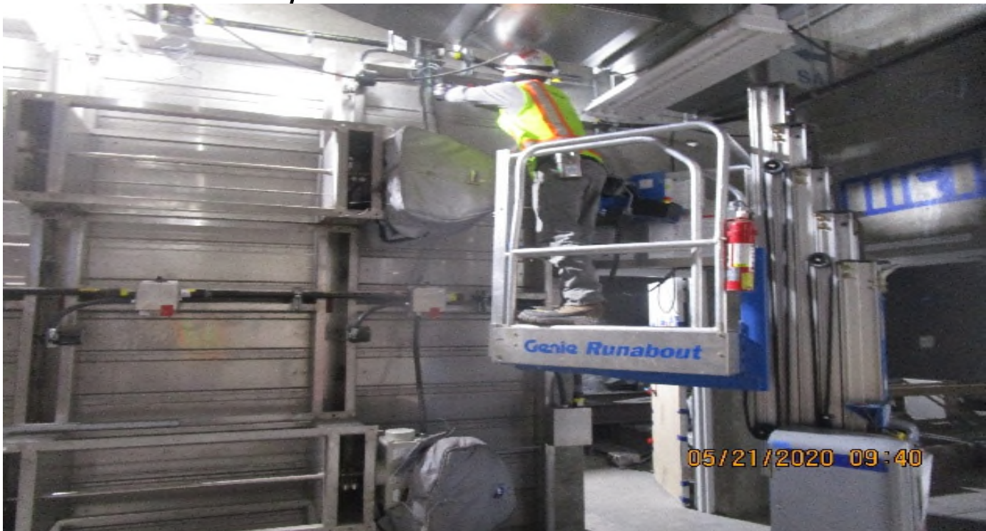
Crenshaw/Vernon - Vernon, Emergency fan (S) C102, pulling (2) #12`s (feeds) & (1) #14 (control) RHW-2 wire at BD-6-301 actuators 1 & 2
