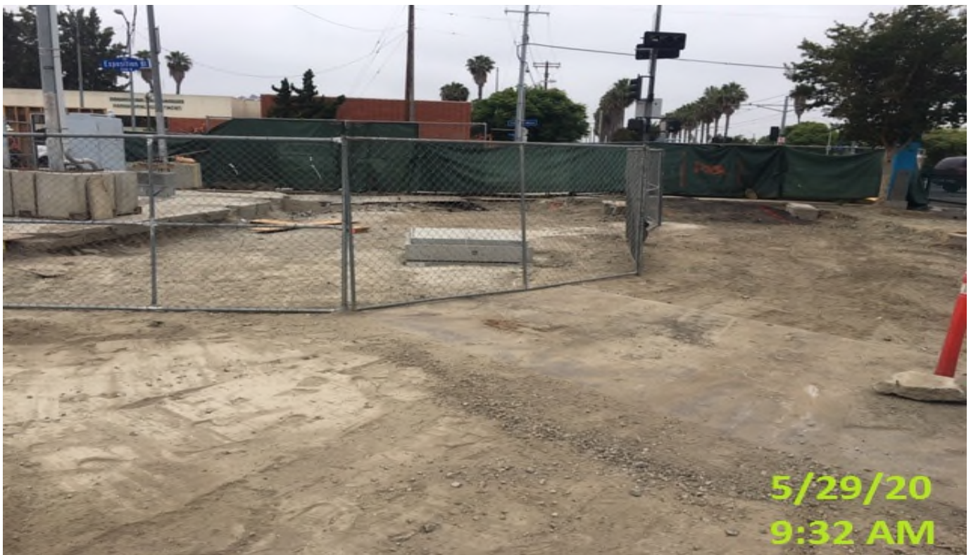
Crenshaw/Expo - WSCC crew resetting fence barricade to protect continued work on tree wells and conduit
