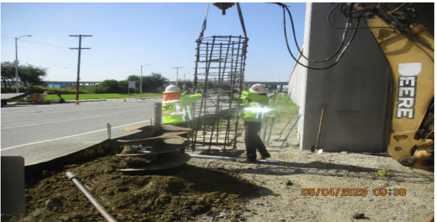
111 th Street – DB Electrical Place cage for SL at S, WCOR of Aviation and 111th.
