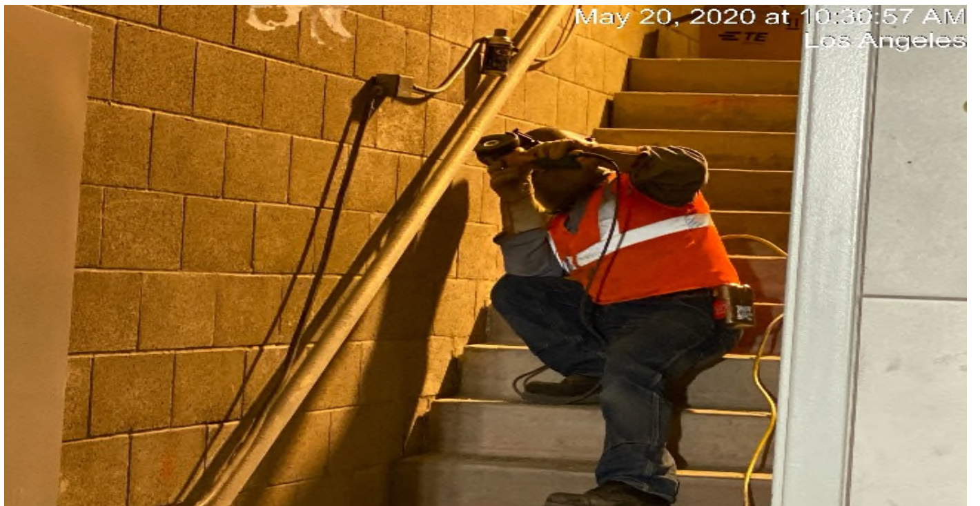
LEIMERT PARK STATION – Continue installing handrails in the south emergency exit stairwell leading into the concourse.
