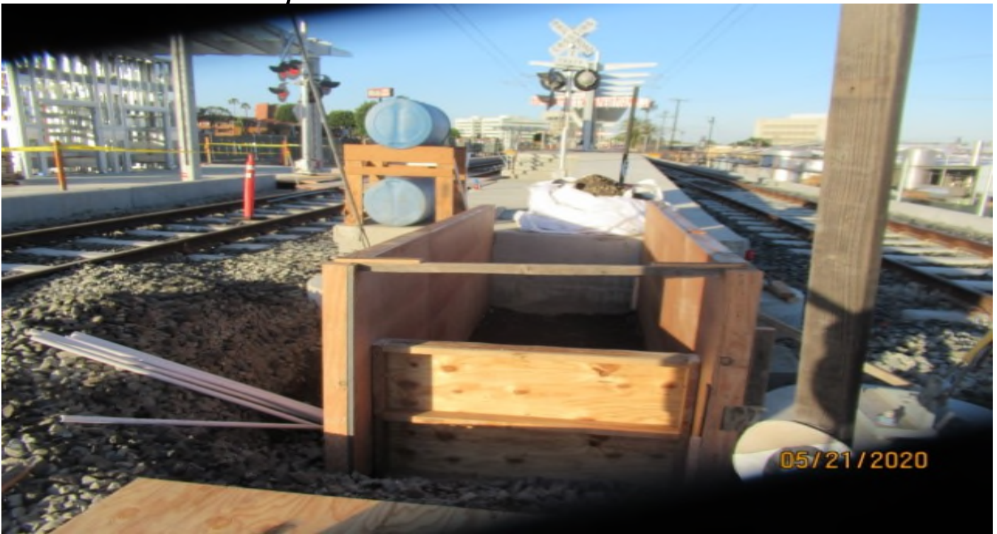
Florence/Brea – WSCC assembling concrete ramp for maintenance access at La Brea station (northend of platform).
