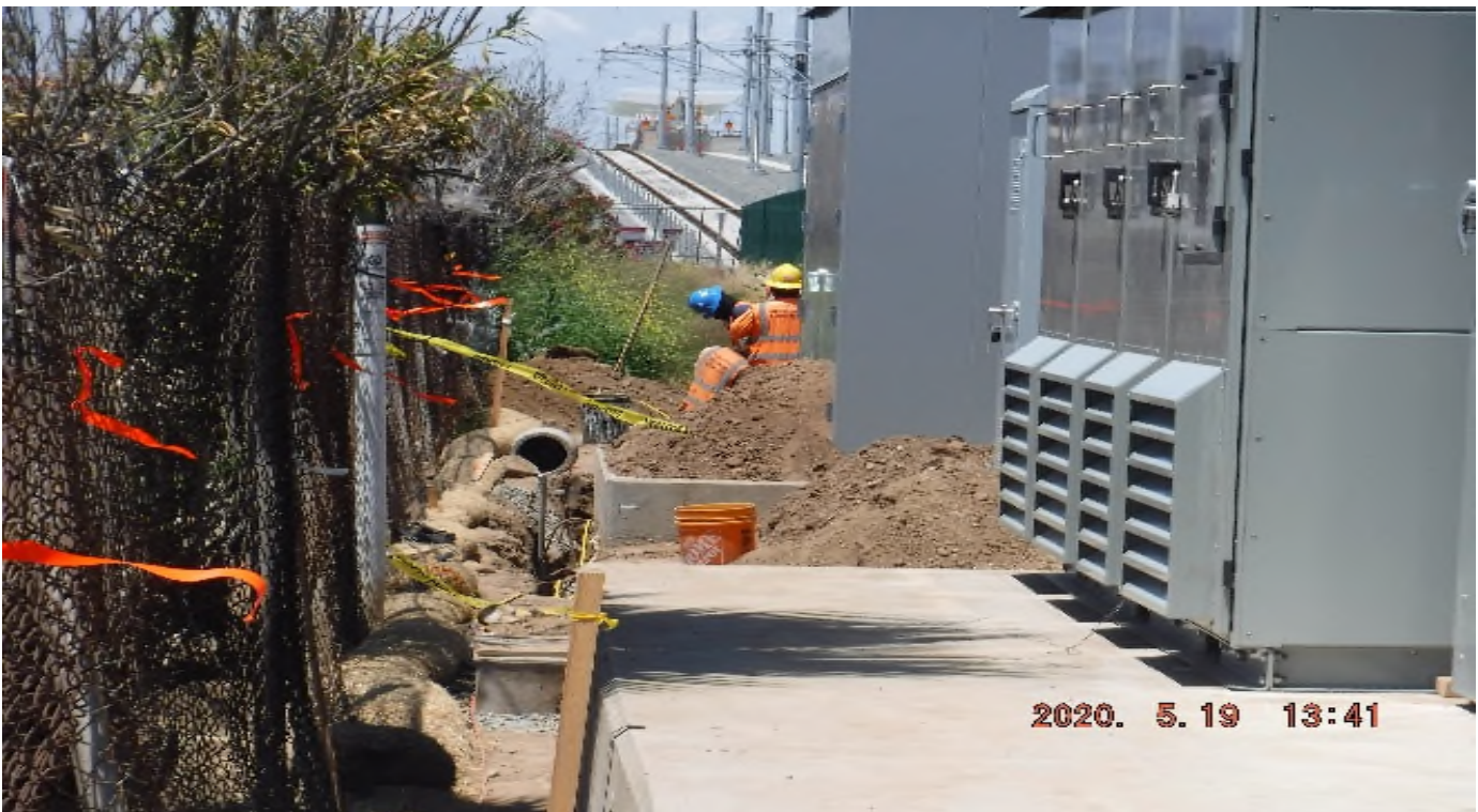
104 th Street - STA 57+00 (TK#3/SB) looking north of 104th St along U1's wall – drainage system work.
