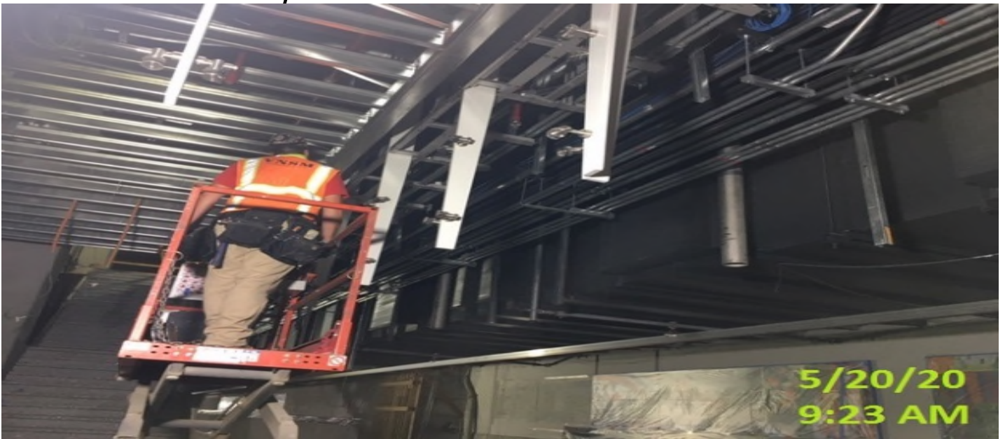
EXPO STATION – Prepping to strip forms for Catch Basin #2 on the northwest section of the plaza.
