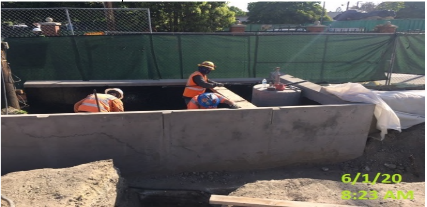
MLK - Continue applying waterproofing membrane sealant for the interior of the planter walls at the plaza level.
