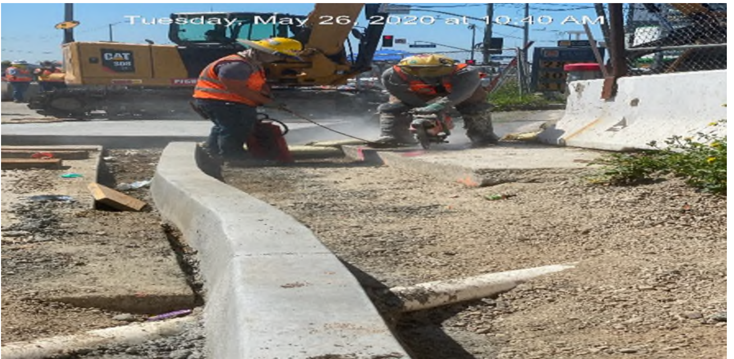
EXPO STATION – Saw cutting existing driveway on southbound Crenshaw Blvd between Exposition Blvd and Rodeo Blvd.
