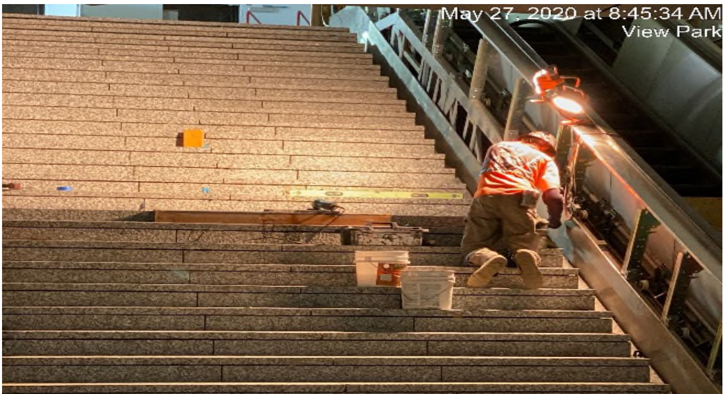
LEIMERT PARK STATION – Continue granite thread and riser installation from intermediate and concourse staircase landings.
