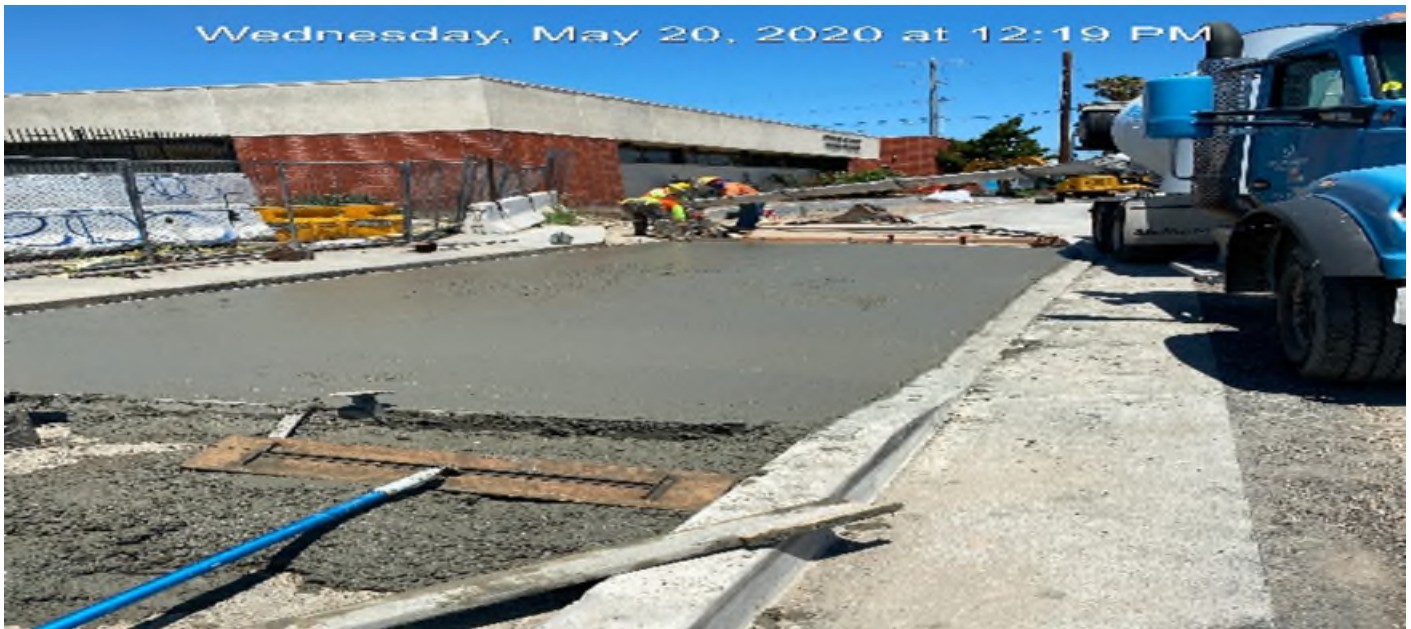
EXPO STATION – Placing concrete for driveway and remaining curb on southbound Crenshaw Blvd between Exposition Blvd and Rodeo Blvd.
