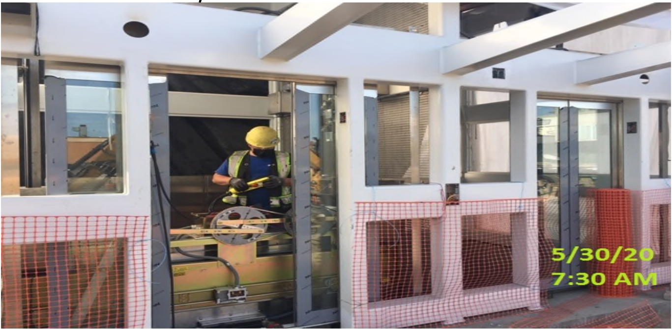
MLK – Wiring limit switches and cab exterior top of Elevator cabs 1&2 at the plaza level.
