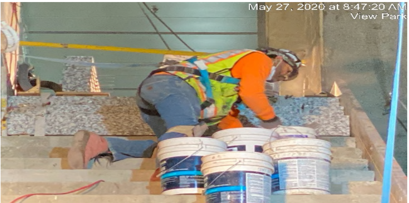
LEIMERT PARK STATION – Began installing granite tread and riser for staircase #4 from concourse to platform level.
