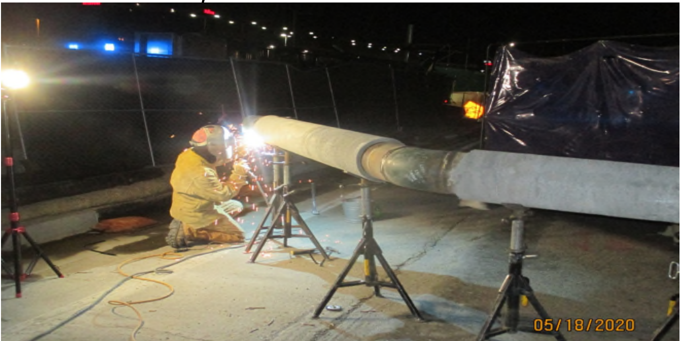
104 th Street - Setting a section of fire line pipe at 104th street
