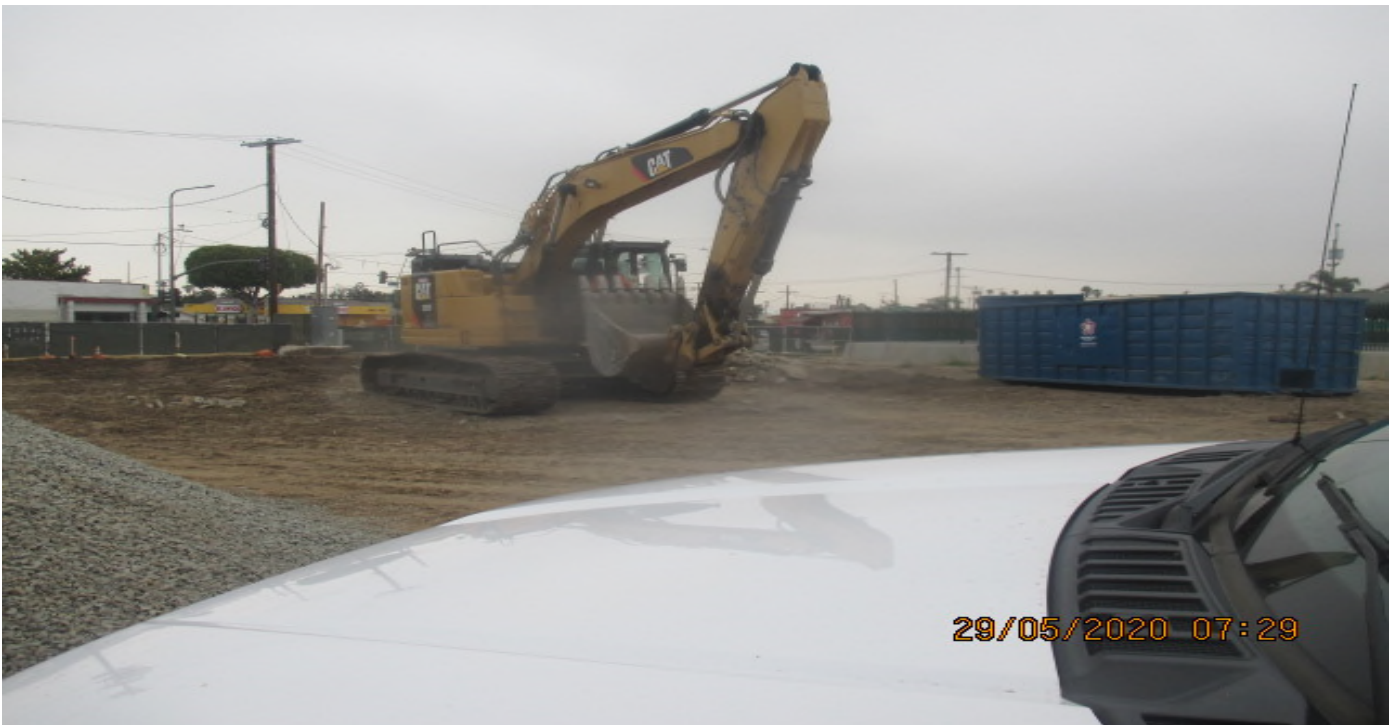
UG3 – Continue excavating the north east section of Victoria Yard for upcoming pavement installation. 5/29/20
