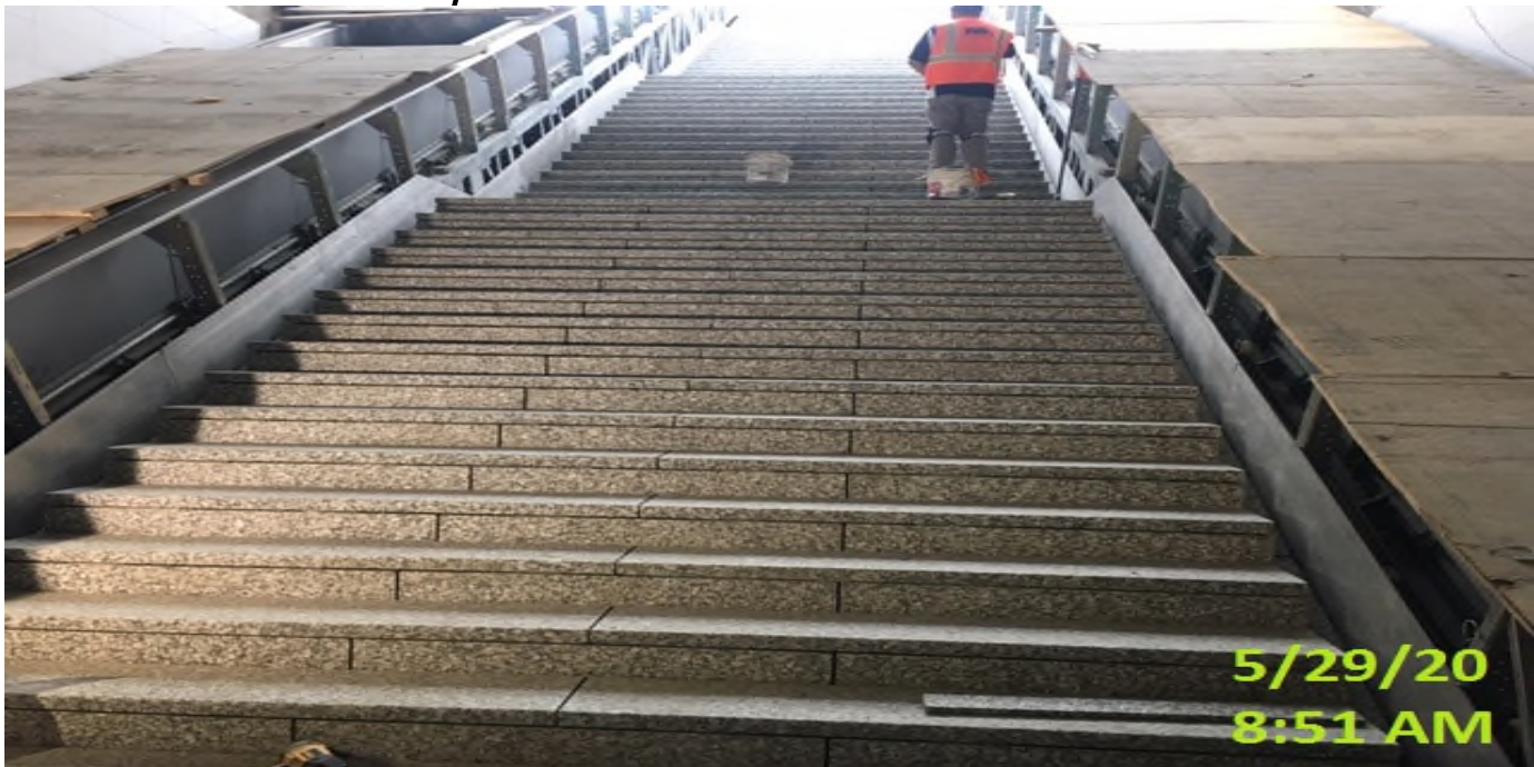
Crenshaw/Expo - WSCC repairing damaged plinths at Expo. Station NB #4 track STA 448+00 (looking north) Rework
