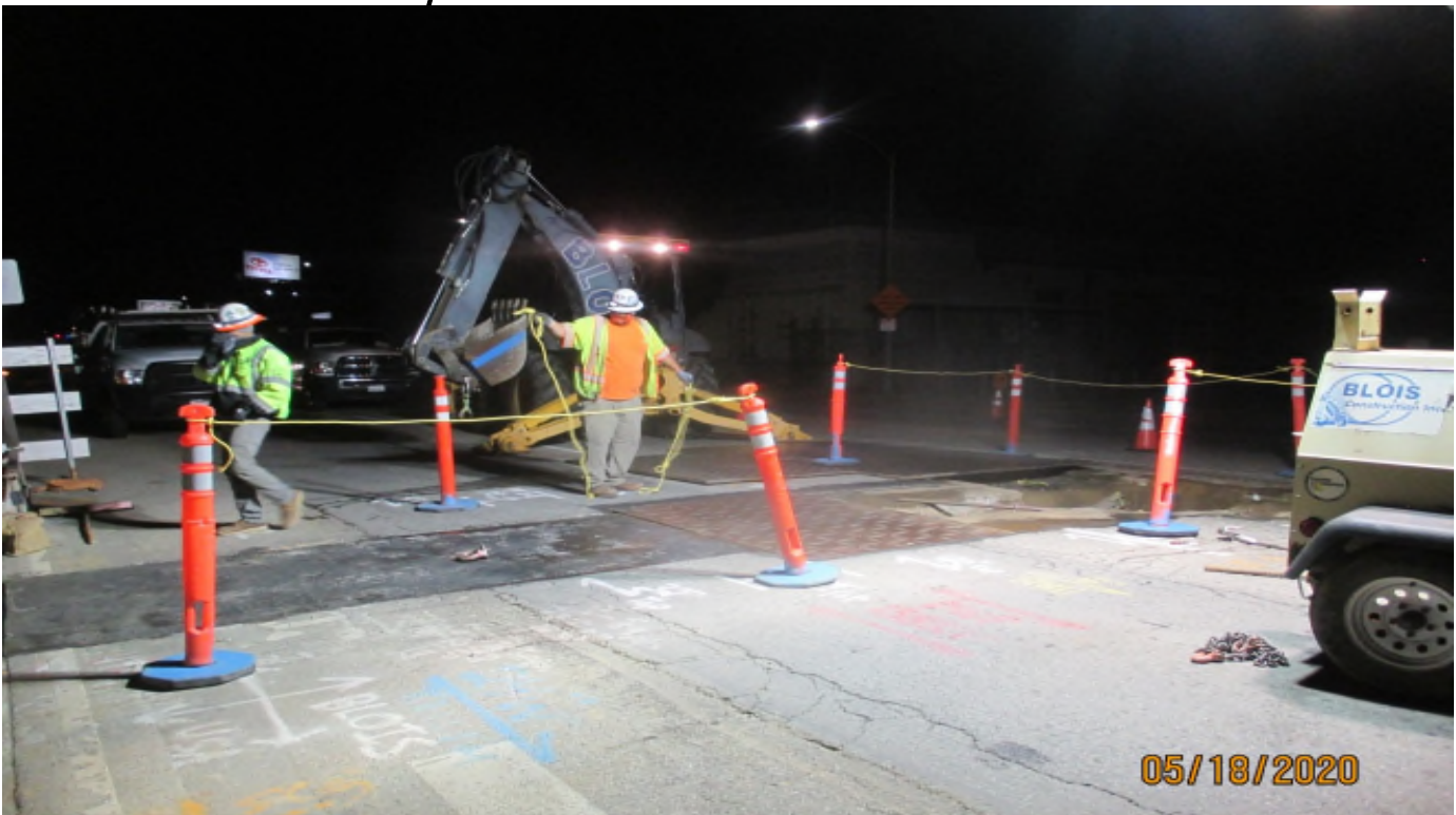
104 th Street - C0988 DH 20200518 Trench plate removal at the 104th street fire line.
