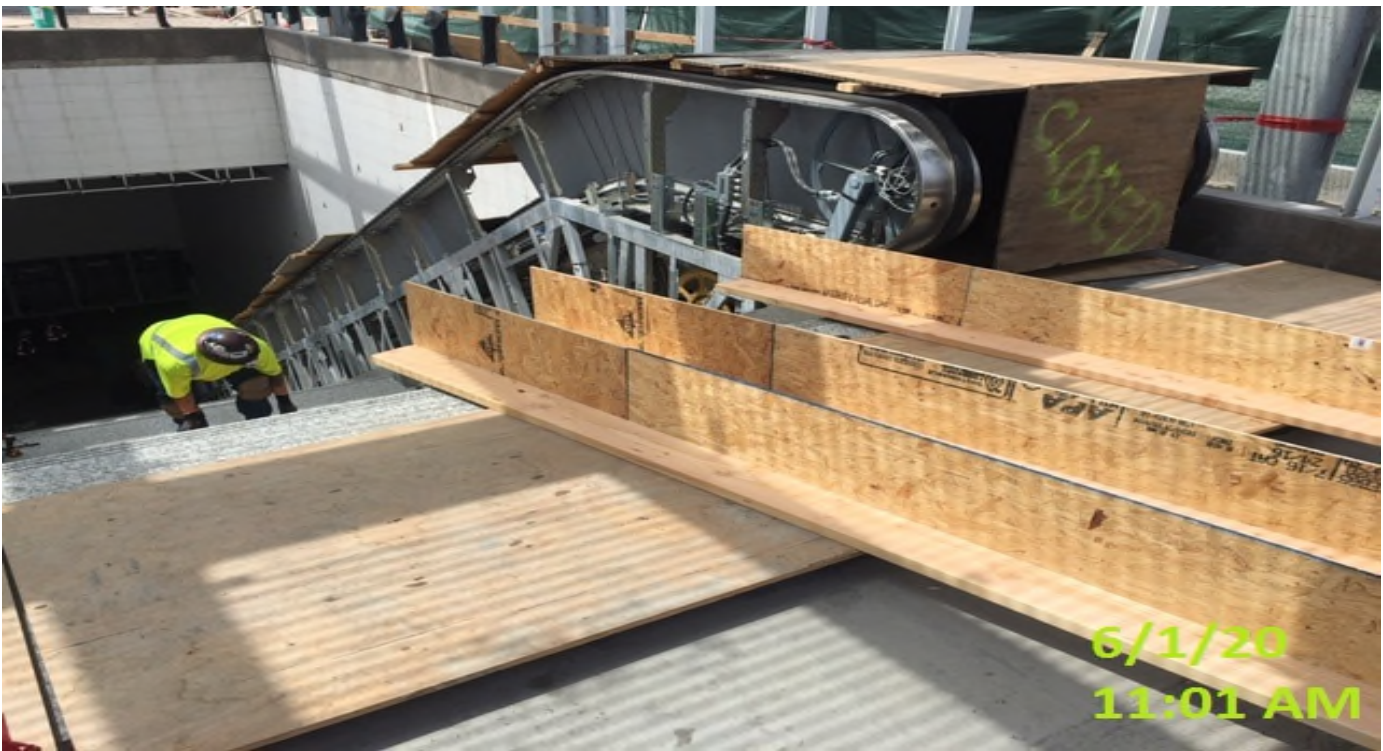
EXPO STATION – Finalizing grouting for the granite risers and treads at the main entrance staircase.
