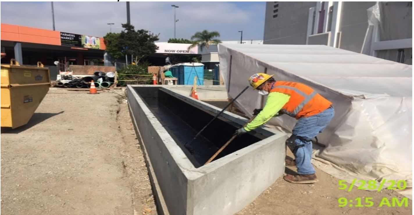
MLK – Continue applying waterproofing membrane sealant for the interior of the planter walls at the plaza level. MLK – WSCC excavating to continue laying 12” HDPE drain line
