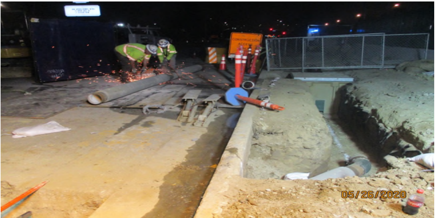
111 th Street – Curb & gutter over-excavation and conduit installation at 111th street. Facing west.
