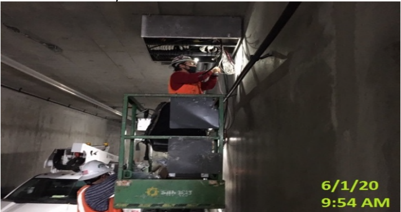
UG3 – Continue splicing permanent power cables along the northbound tunnel at Sta 311+34.
