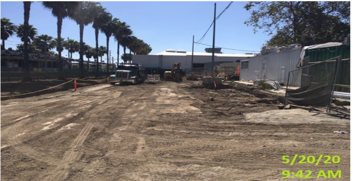
EXPO STATION – Continue excavation/grading for upcoming top soil placement on the north side of the plaza.
