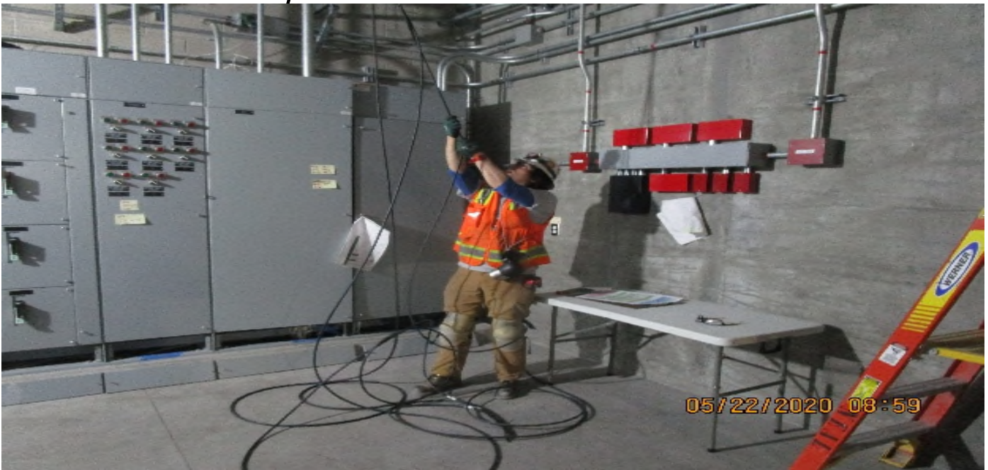
Crenshaw/Vernon - Vernon, Aux Power (S) C110, begin re-pulling 2 pair #14 interlocking between MCC2/S CIC2/S to PX1/S & PX2/S
