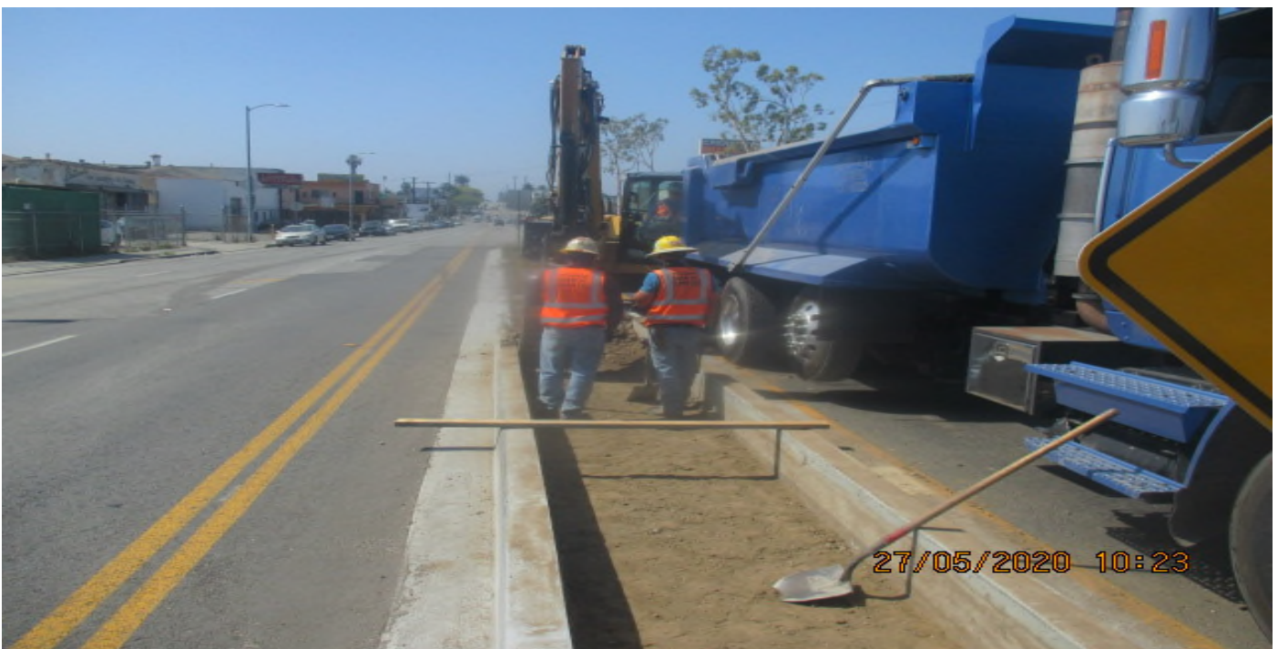
UG3 – Excavating for median cobble installation on the median island south of 67th St and Crenshaw Blvd. 5/27/20
