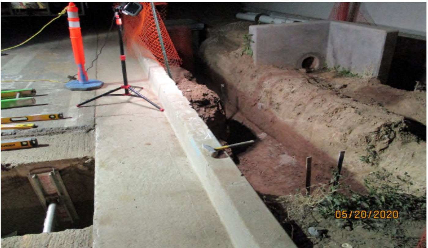
104 th Street - Fire line trench where the 2 45 degree connections will go on 104th street.
