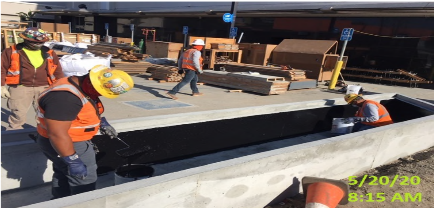
MLK Station - MLK – Began applying waterproofing membrane sealant for the interior of the planter walls at the plaza level.
