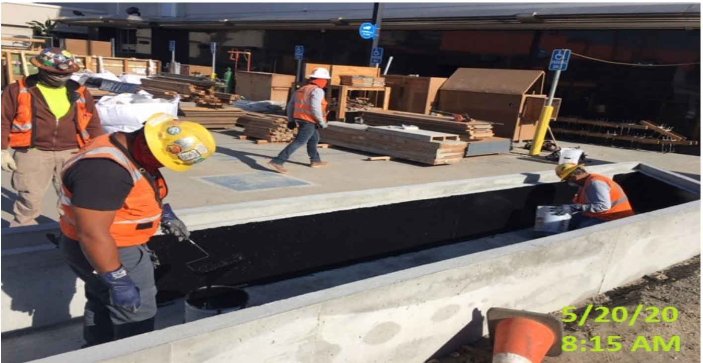
Crenshaw/MLK - MLK – WSCC carpenters applying waterproof sealant on insides of planter walls.
