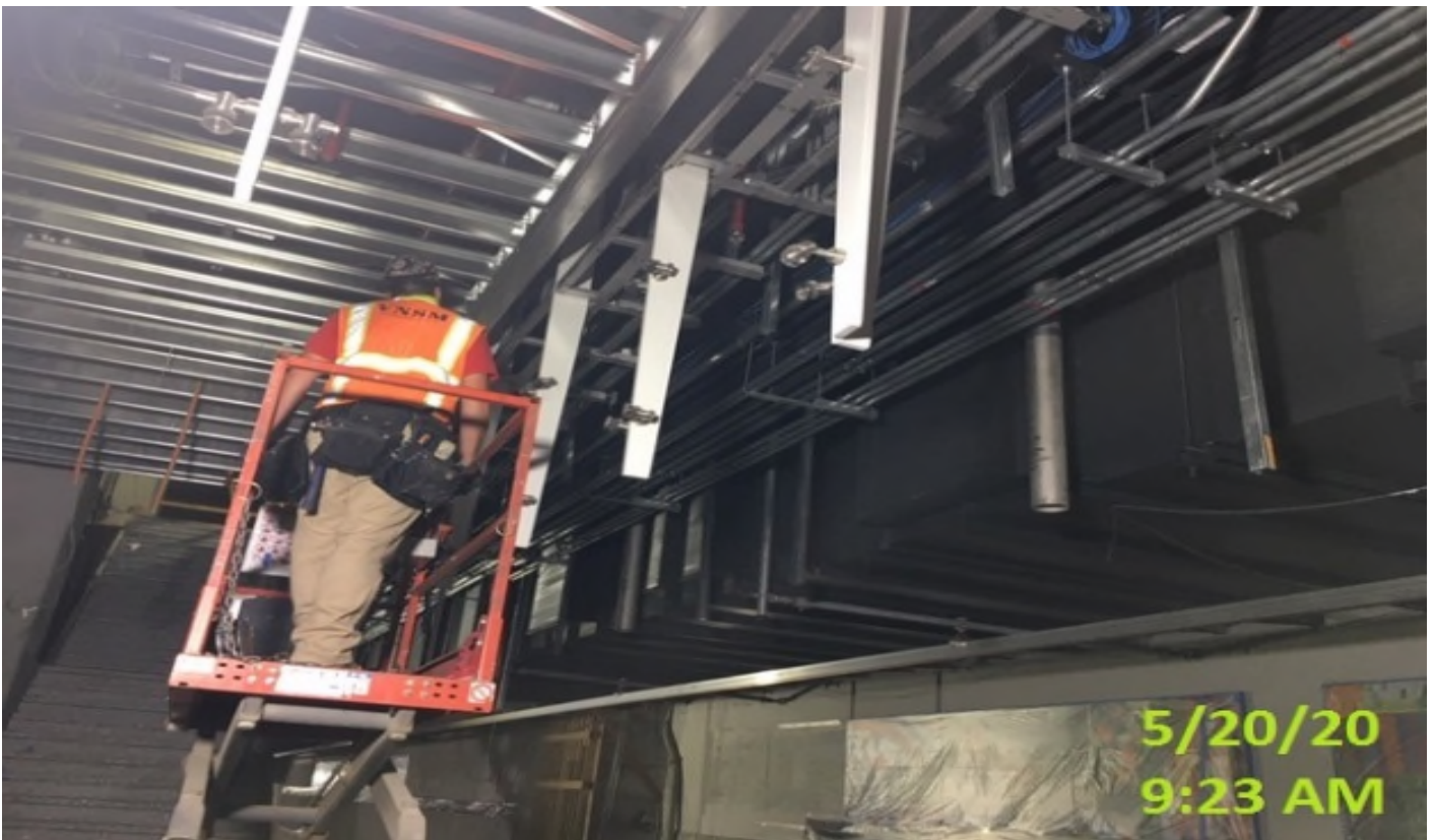
Crenshaw/Expo - VNSM installing clad panels in smoke screen area of platform level.
