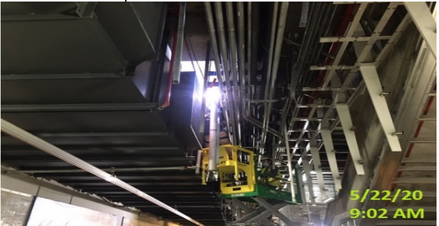
EXPO STATION – Welding sleeve joints for the supports posts for the platform edge lighting.
