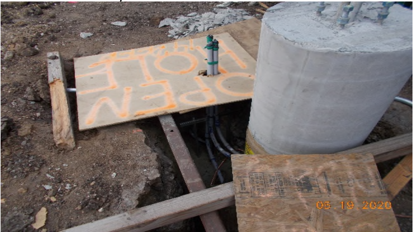
60 th Street - View of light pole and conduits ready for vault. 60th street.
