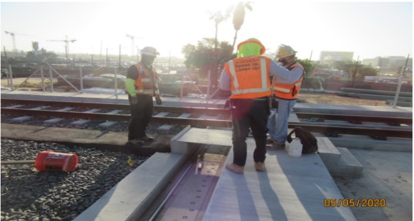
Aviation/Century – WSCC QC & concrete foreman going over open item punch list, Activity #1498 on Century/Aviation bridge (looking east) rework
