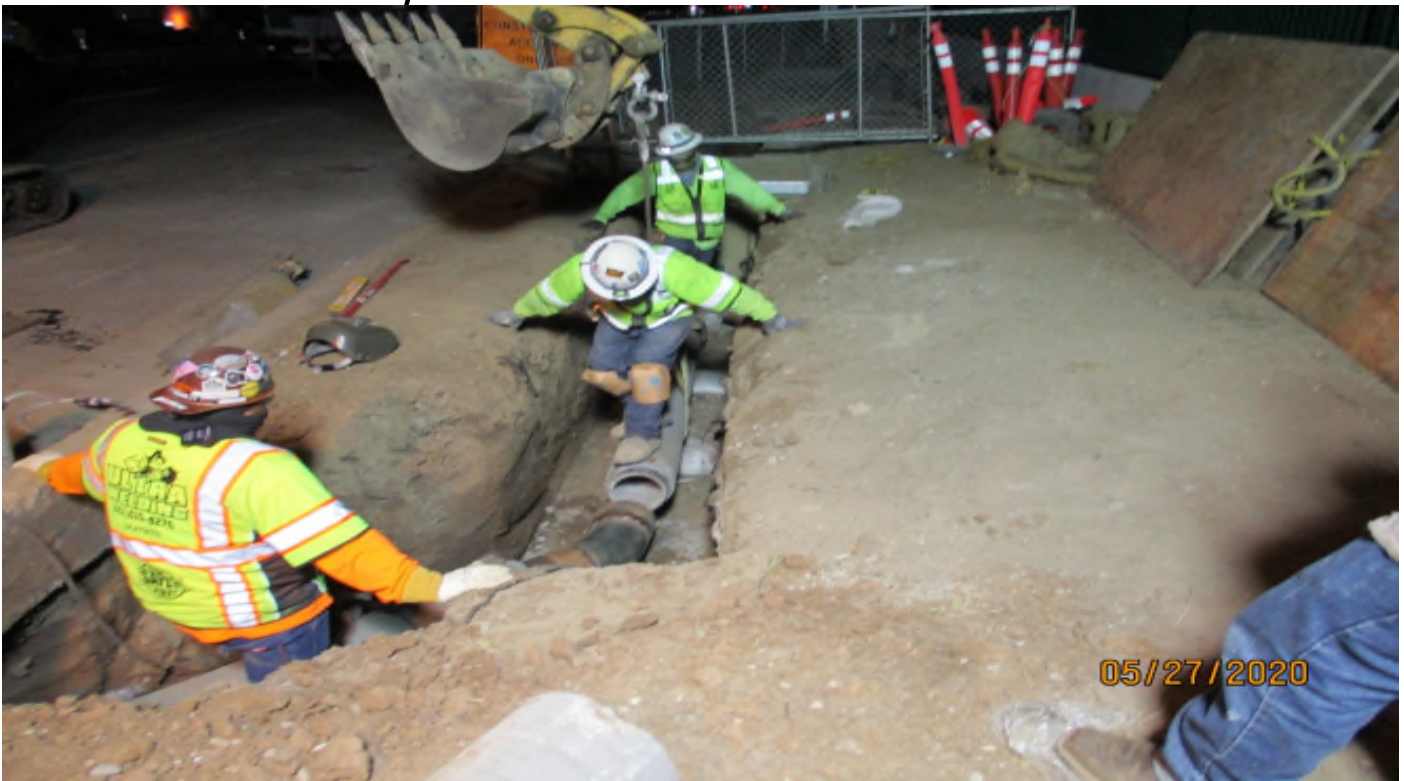
111th Street – Setting a section of fire line pipe at 111th street.
