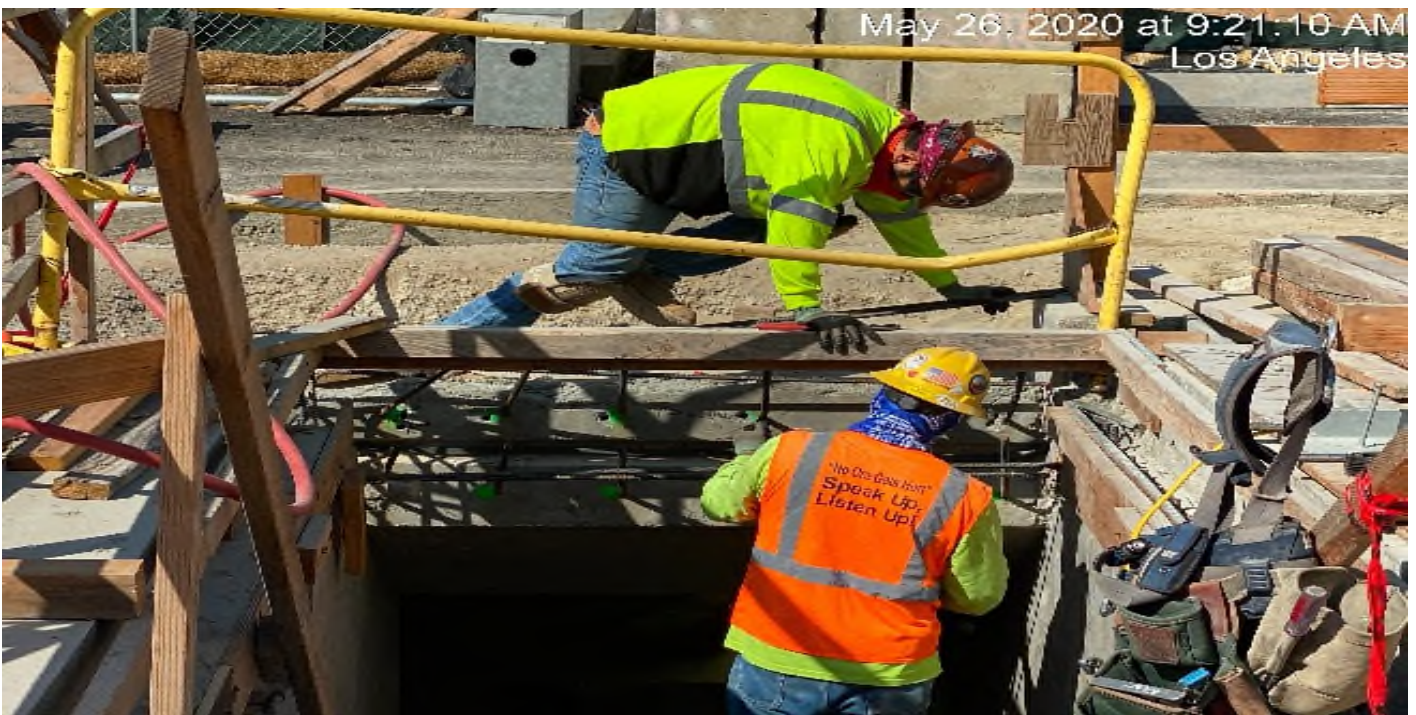
LEIMERT PARK STATION – Continue drilling and doweling for the south emergency exit hatch doors at the plaza level.
