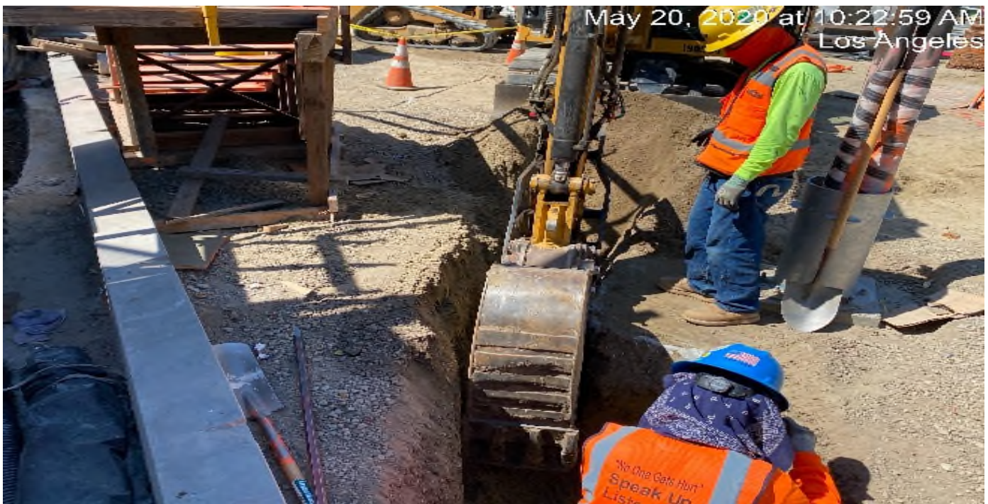
LEIMERT PARK STATION – Excavating/trenching for conduit installation on the east side of the plaza level.
