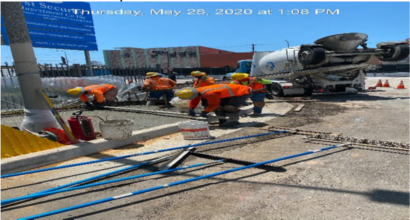
LEIMERT PARK STATION – Placing concrete for new ADA ramp and sidewalk on the southeast corner of 46th St and Crenshaw Blvd.
