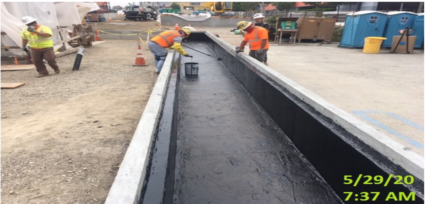
MLK - Continue applying waterproofing membrane sealant for the interior of the planter walls at the plaza level.
