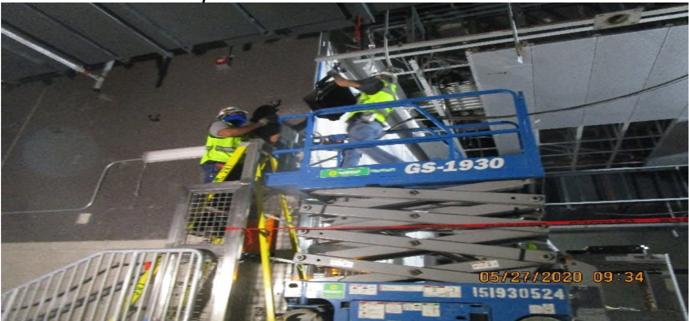
LEIMERT PARK STATION – Began installing flashing hand signal displays above the north and southbound end gates at the south end of the platform level.
