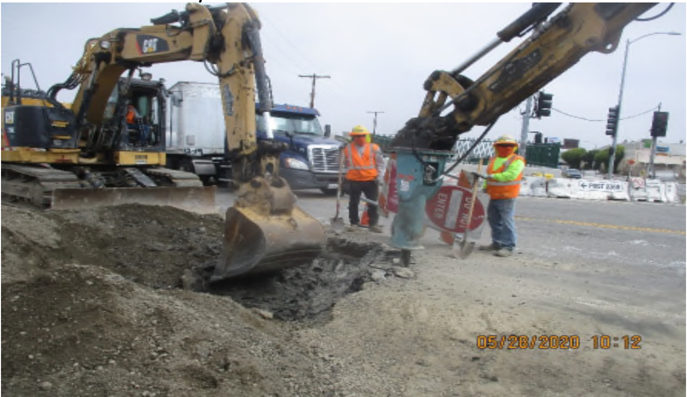
Aviation/Century – WSCC Continued Making removals and C&G Grade at 104th and Aviation.
