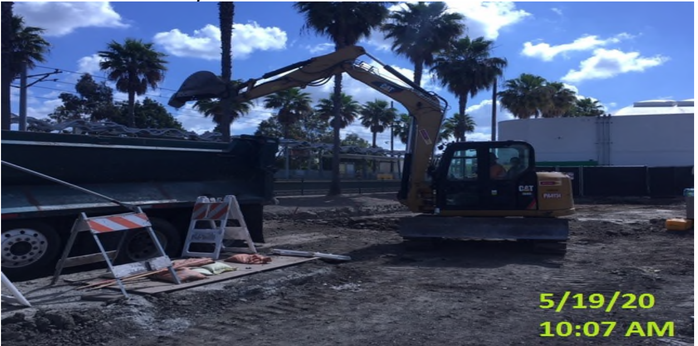
EXPO STATION – Resume excavation/grading for upcoming top soil placement on the north side of the plaza.
