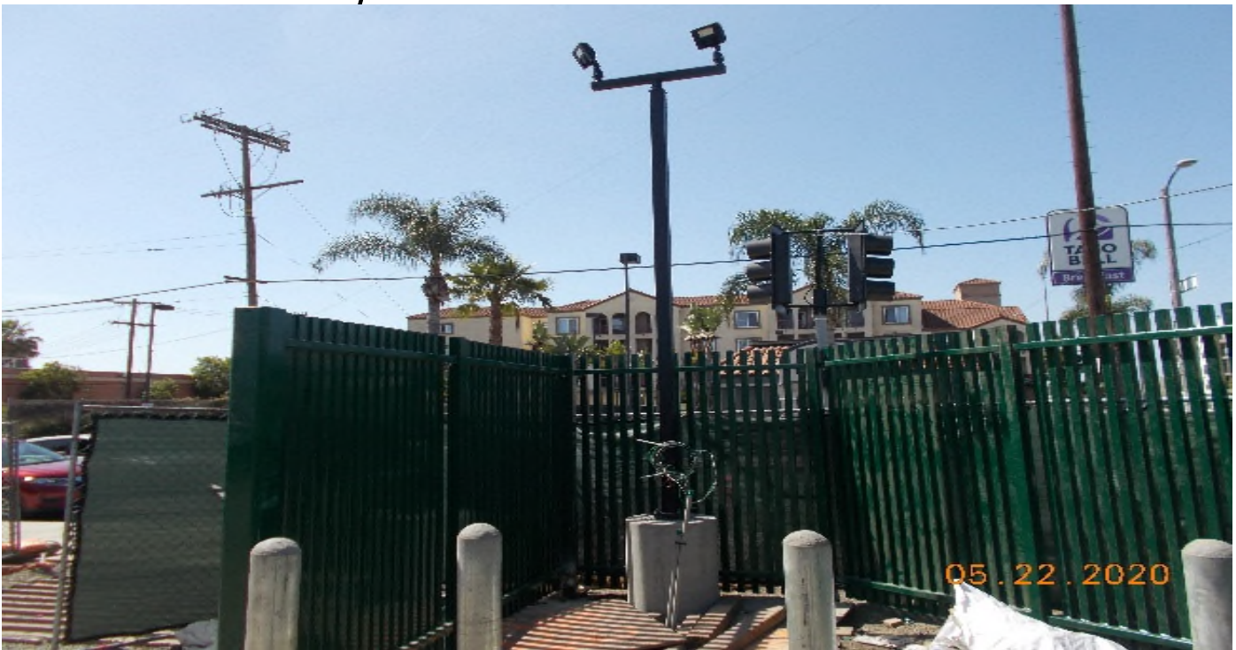
PARK MESA – Completed light pole foundation at the northeast corner of TPSS#7 on 60th St & Crenshaw Blvd.
