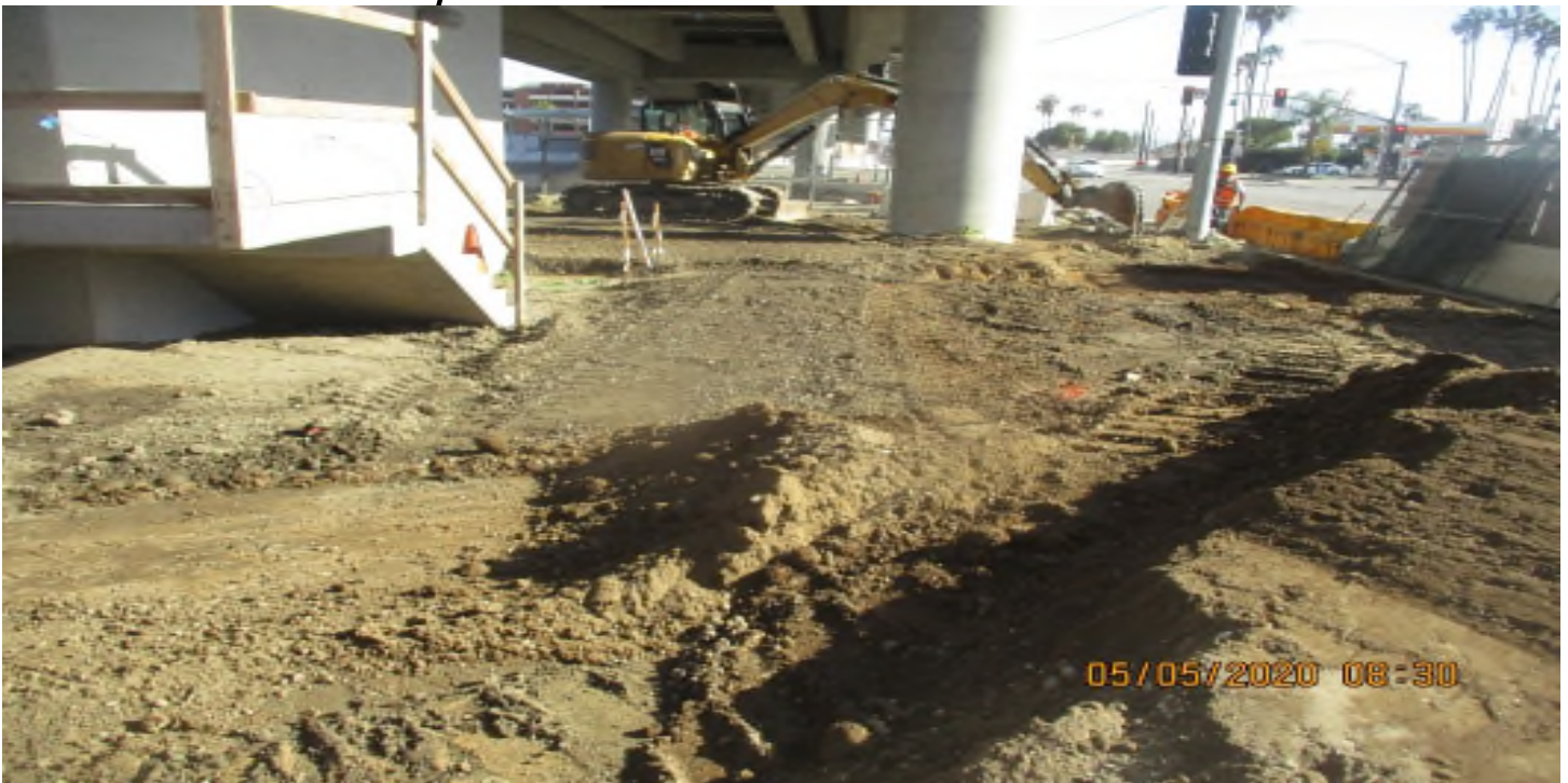
Aviation/Century – WSCC Make SWK and land scape grade Century and Aviation under bridge.
