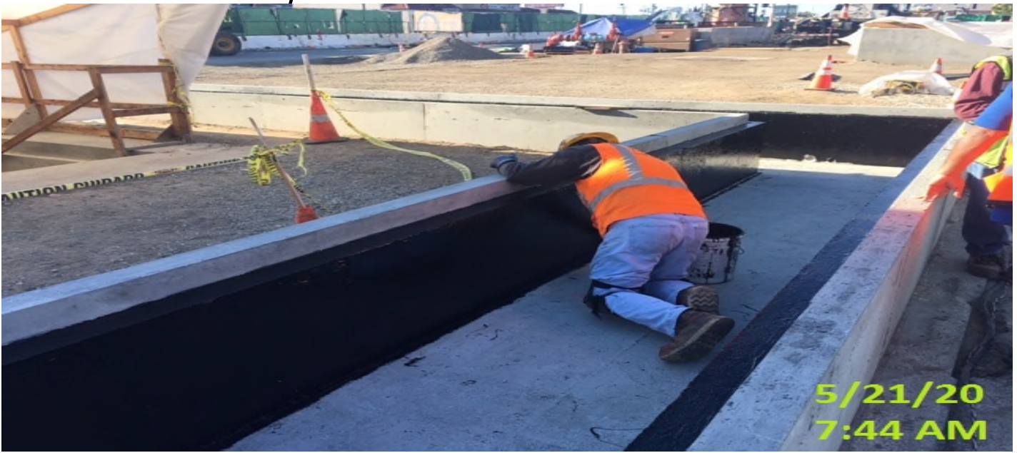
MLK Station - Continue applying waterproofing membrane sealant for the interior of the planter walls at the plaza level.
