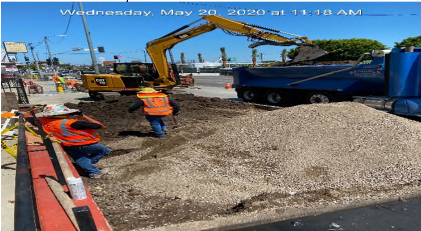
LEIMERT PARK STATION – Placing backfill for new sidewalk installation on southbound Crenshaw Blvd between Vernon Ave and 43rd Pl.
