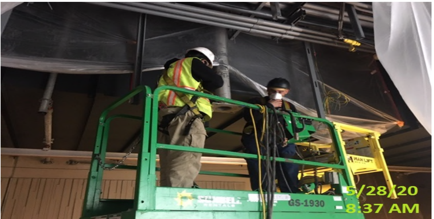
EXPO STATION – Continue welding upper plates to the supports posts for the platform edge lighting.
