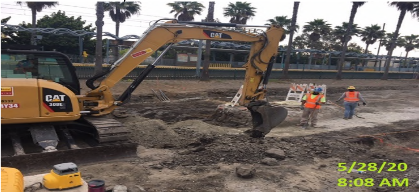
EXPO STATION – Continue excavation/grading for upcoming top soil placement on the north side of the plaza.
