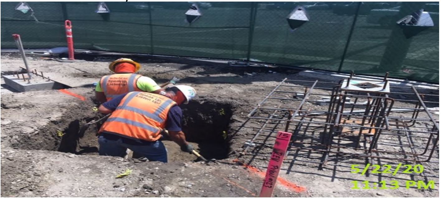
MLK, Digging for upcoming grand pylon foundation at the northeast corner of the plaza level.
