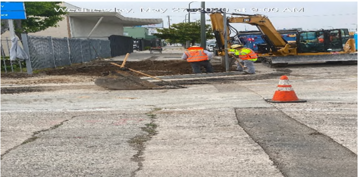
LEIMERT PARK STATION – Excavating for the installation of a street light foundation on the southeast corner of 46th St and Crenshaw Blvd.
