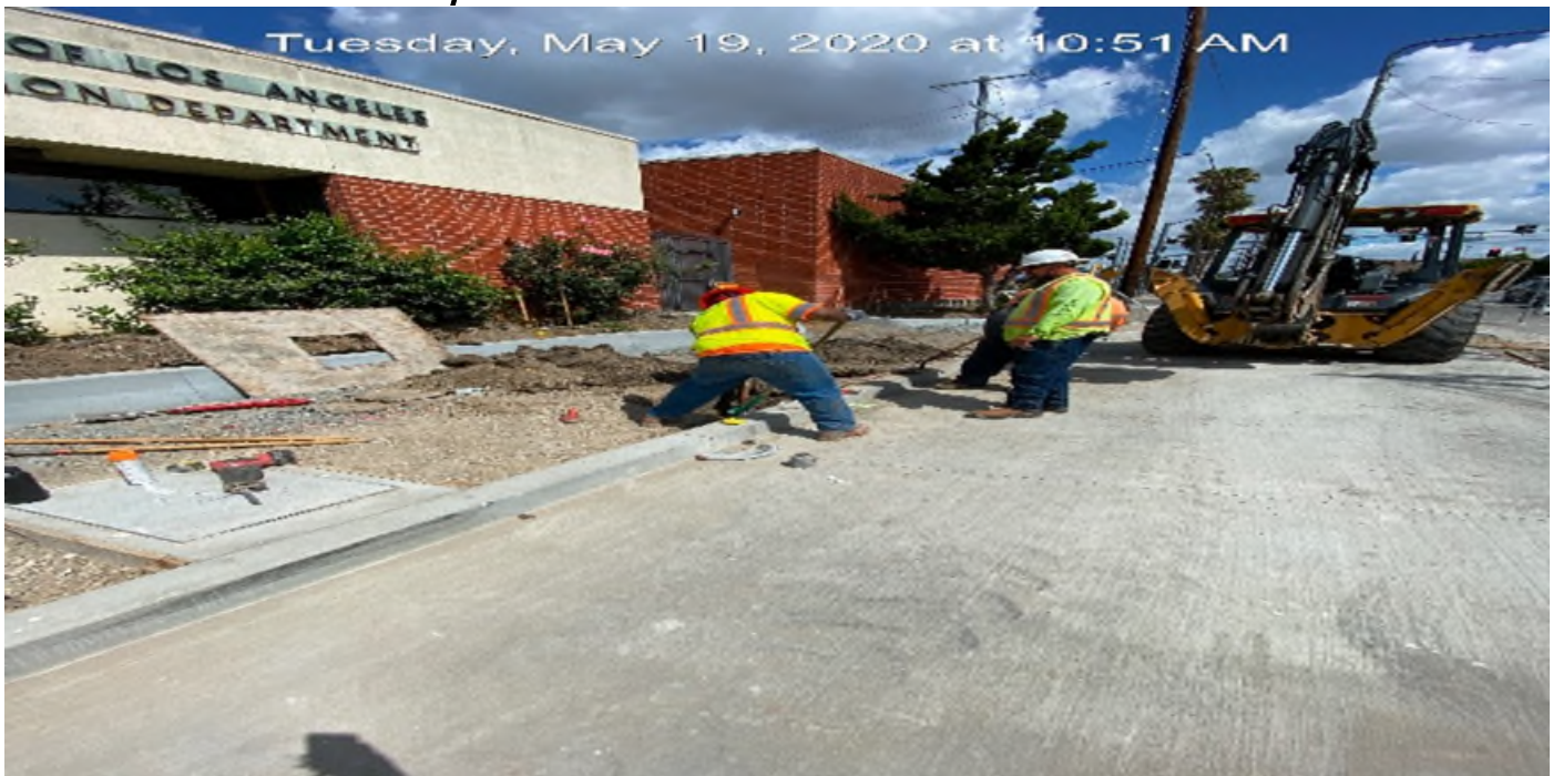
EXPO STATION – Excavating for street light foundations and pull boxes on southbound Crenshaw Blvd between Exposition Blvd and Rodeo Blvd.
