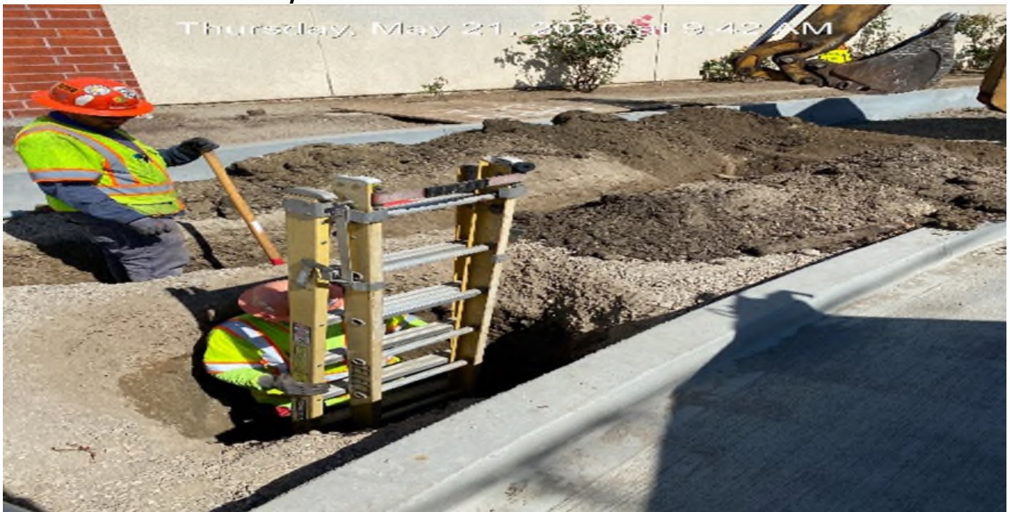
EXPO STATION – Continue excavating for street light foundations and pull boxes on southbound Crenshaw Blvd between Exposition Blvd and Rodeo Blvd.
