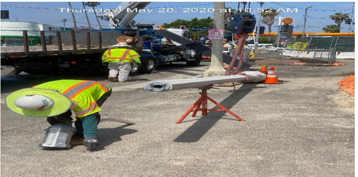
EXPO STATION – Installing concrete street light poles on westbound Rodeo Blvd between Crenshaw Blvd and Bronson Ave.
