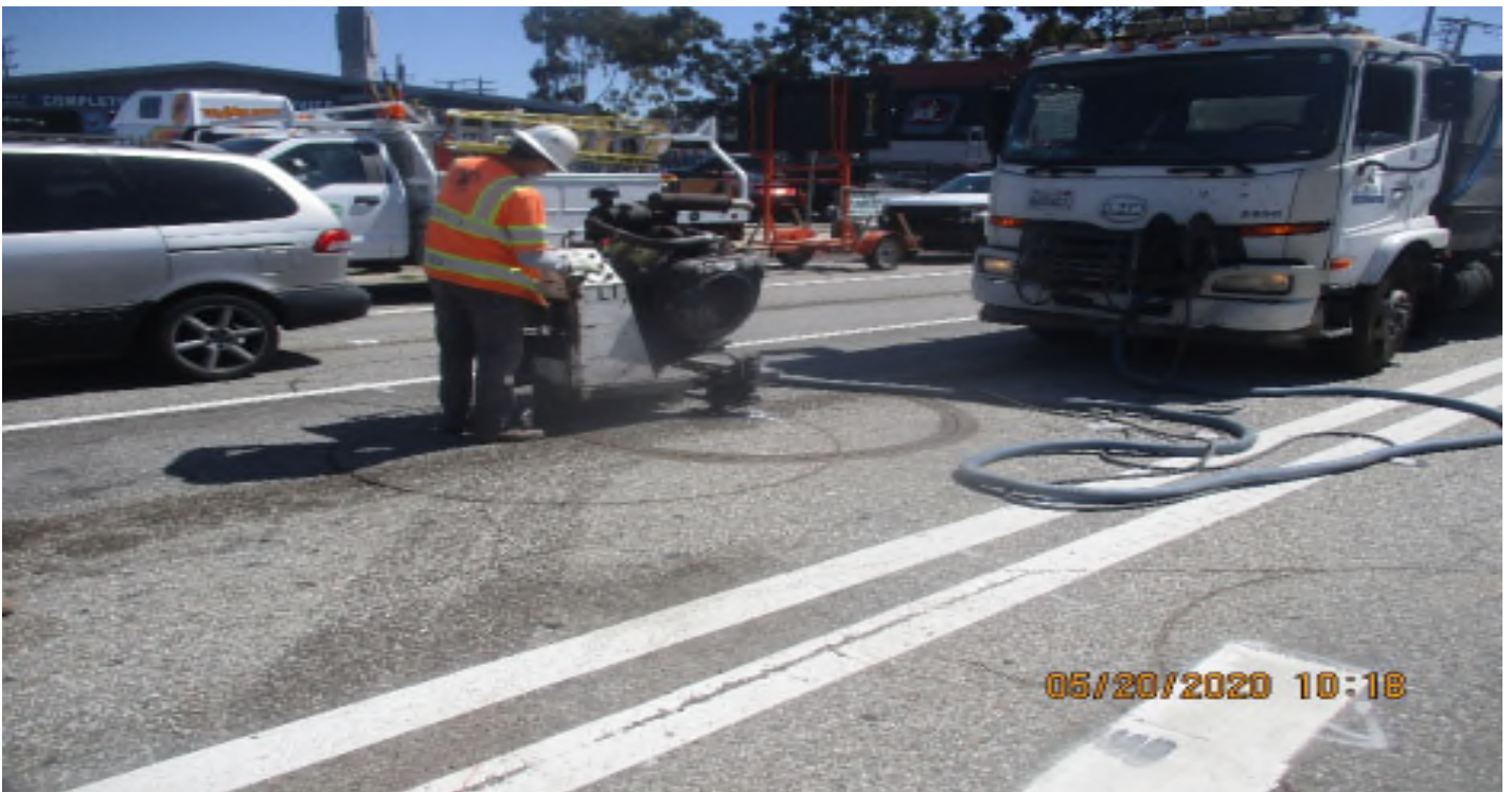
Manchester Bridge – GRSI Saw cut loops at Manchester intersection.
