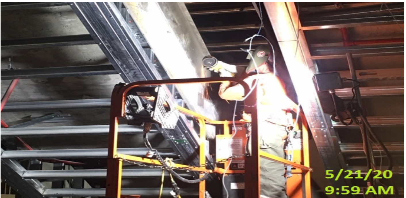
EXPO STATION – Cutting/grinding for handrail post installation for staircase #3 from concourse to platform level.
