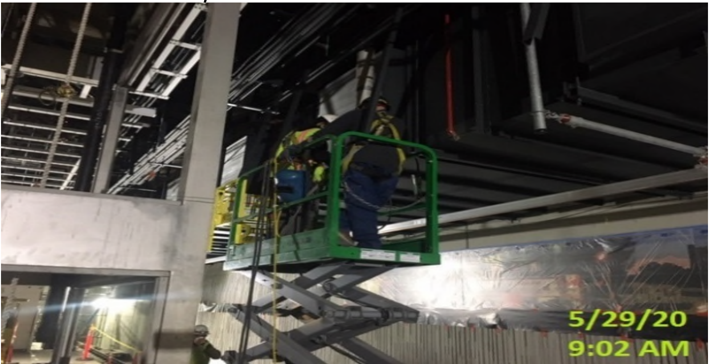
EXPO STATION – Continue welding upper plates to the supports posts for the platform edge lighting.
