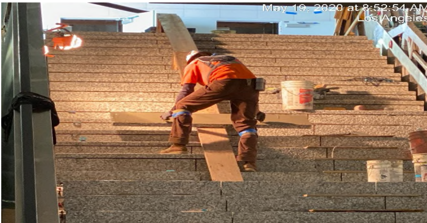
LEIMERT PARK STATION – Continue granite thread and riser installation from intermediate and concourse staircase landings.
