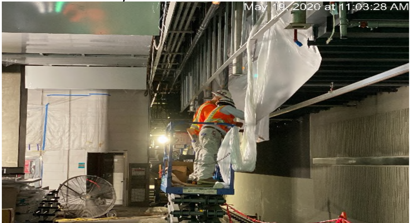
LEIMERT PARK STATION – Continue applying finish paint to the ceiling conduits at the platform level.
