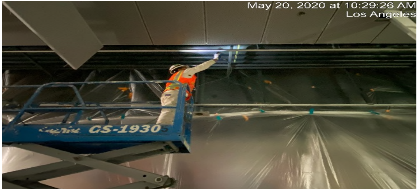
LEIMERT PARK STATION – Continue applying finish paint to the ceiling conduits at the platform level.
