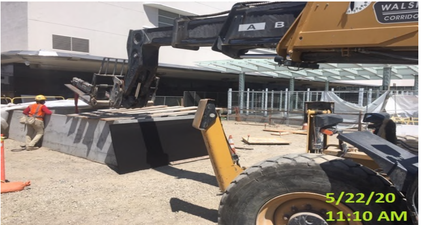
MLK - Installing anchors for the steel ladders inside the north vent shaft at the plaza level.
