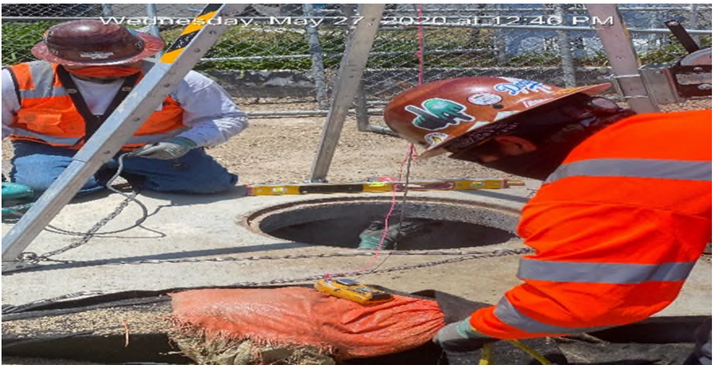
EXPO STATION – Continue installing steel steps for Catch Basin #16 on southbound Crenshaw Blvd between Exposition Blvd and Rodeo Blvd.
