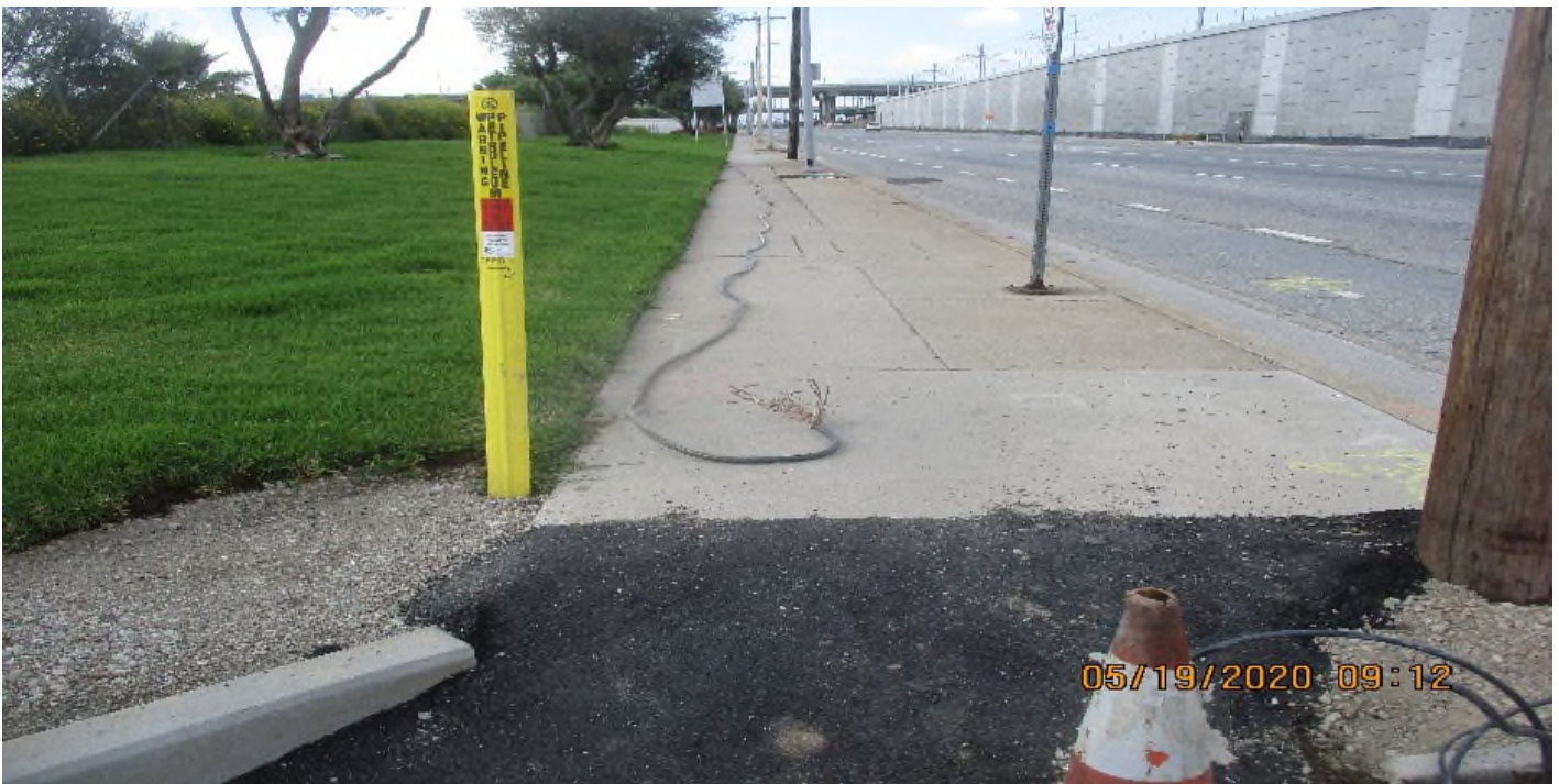
111th Street – DB Electric Removed loop cable at N,B Aviation at 111Th St.
