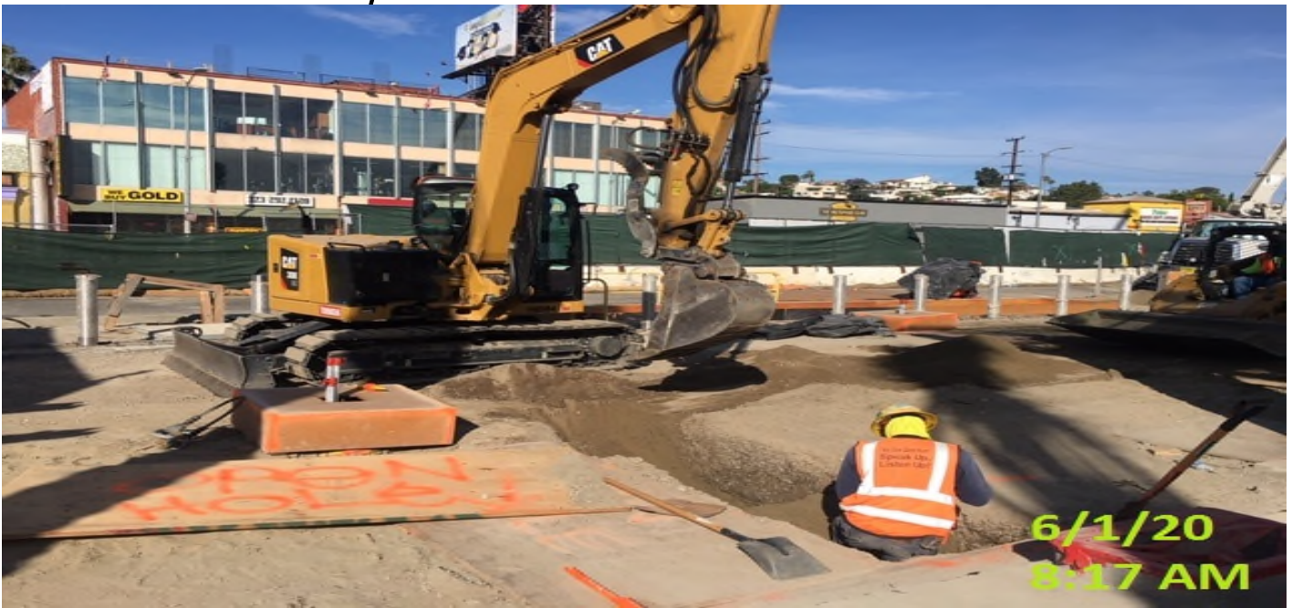
LEIMERT PARK STATION – Continue excavating/trenching for underground conduit installation for landscape lighting for palm trees and canopy at the south side of the plaza level.
