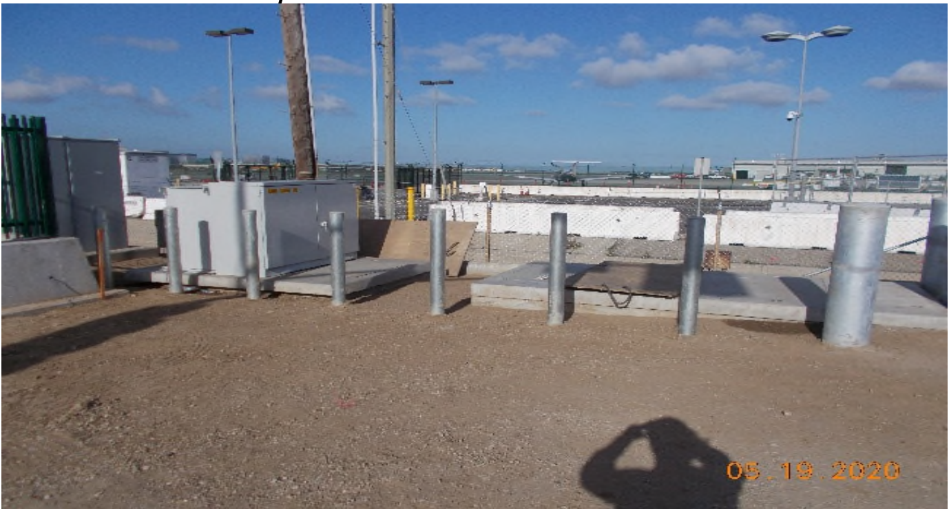
104 th Street - West view of DWP transformer. 104 th
