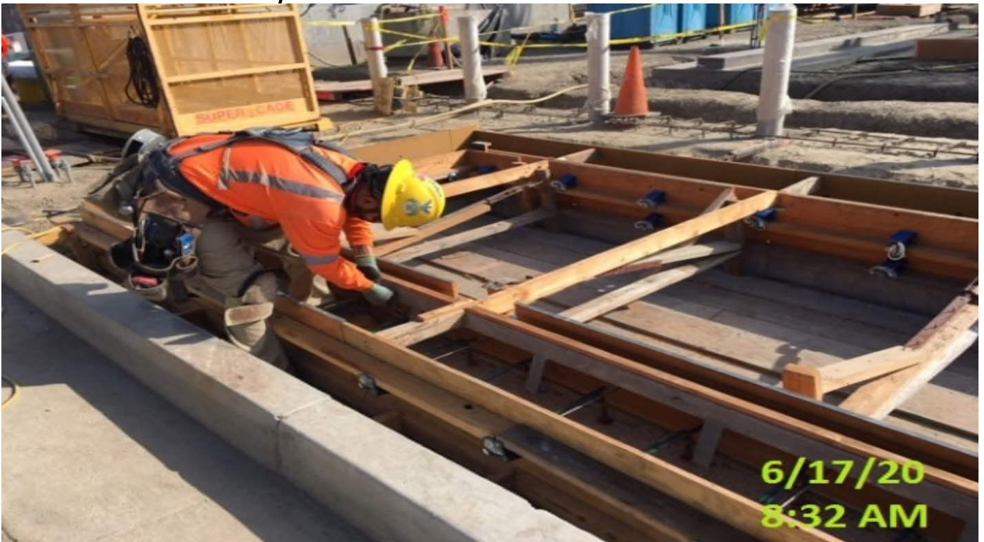
LEIMERT PARK STATION – Continue building formwork for the air exhaust shaft at the plaza level.
