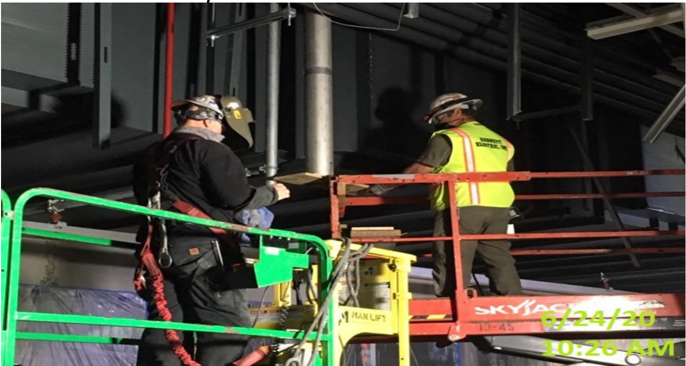
EXPO STATION – Continue welding and plumbing southbound edge light support poles along the platform level.
