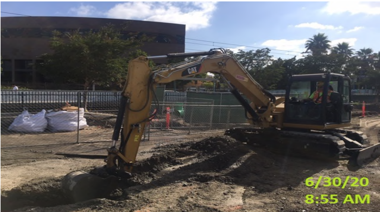
EXPO STATION – Continue excavating wells for palm tree installation throughout the plaza level.
