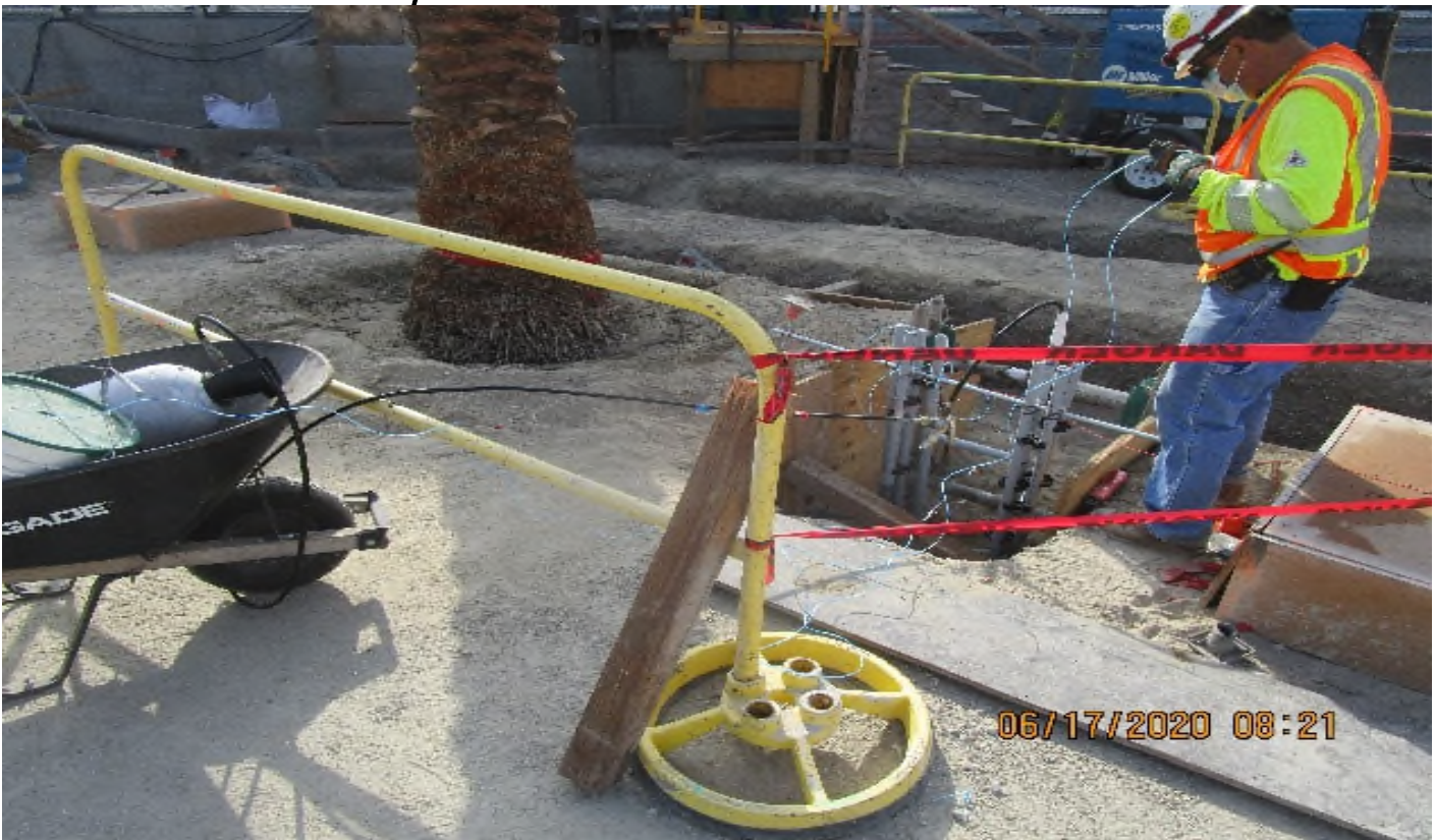
LEIMERT PARK STATION – Continue underground conduit installation for landscape lighting and utilities at the plaza level.
