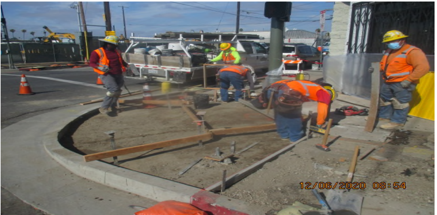
UG3 – Grading for sidewalk installation for a section of the Victoria Cul-de-sac radius. 6/17/20
