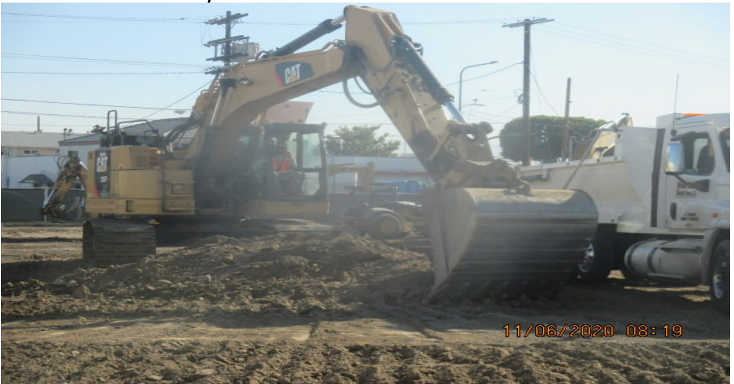
UG3 – Continue grading the north east section of Victoria Yard for upcoming pavement installation. 6/11/20
