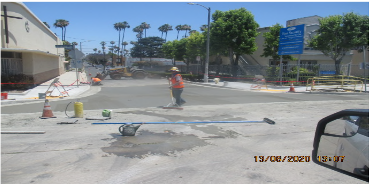
LEIMERT PARK STATION – Placed new concrete pavement for the intersection of 46th St and Leimert Blvd. 6/13/20
