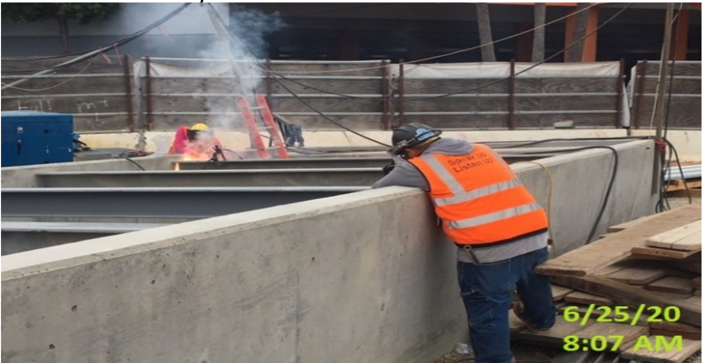
MLK STATION – Continue installing beams for steel grating for the south air exhaust vent shaft at the plaza level.
