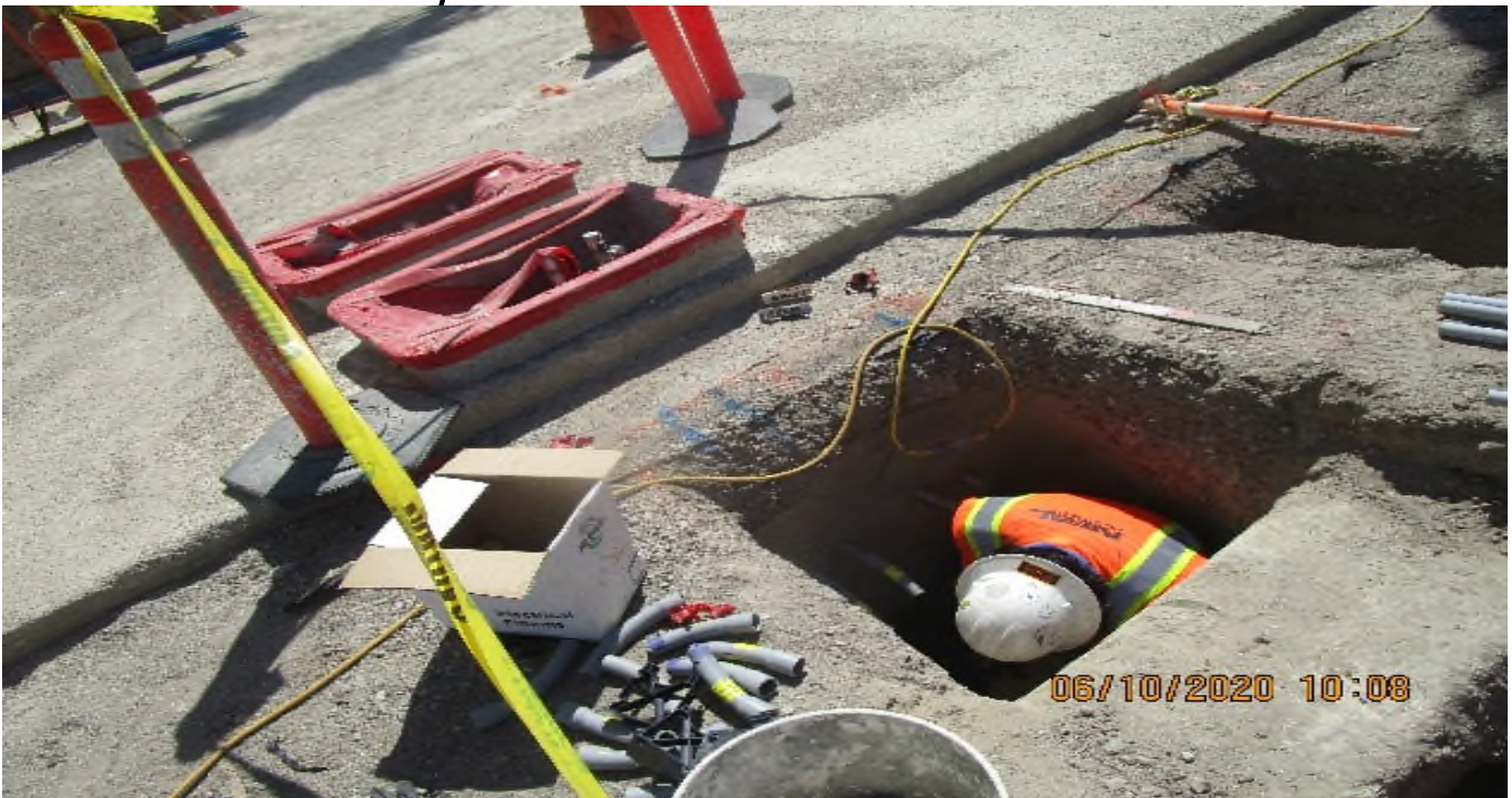
LEIMERT PARK STATION – Continue underground conduit installation for landscape lighting and utilities at the plaza level.
