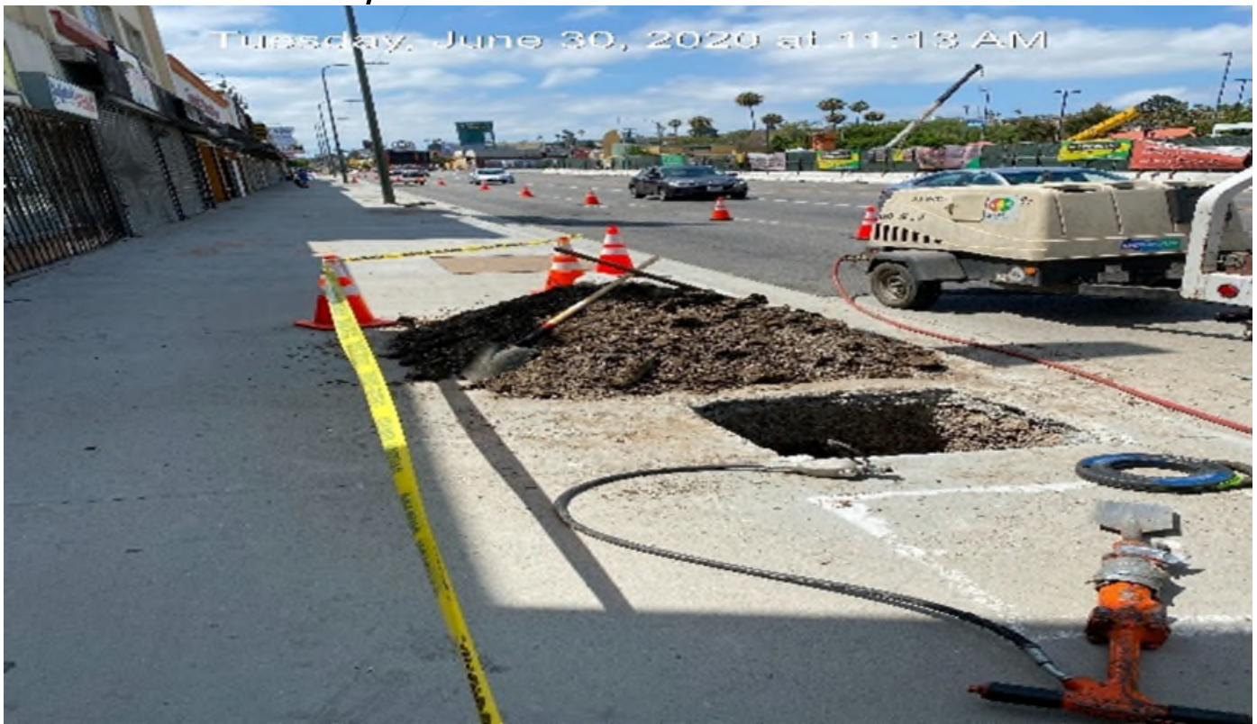
MLK STATION – Excavating for new pedestrian signal head foundations on Crenshaw Blvd between Stocker St and MLK Blvd.
