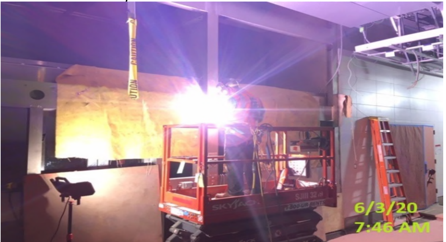
MLK – Began welding the fascia mesh screen panels to Elevators 3&4 at the concourse level.
