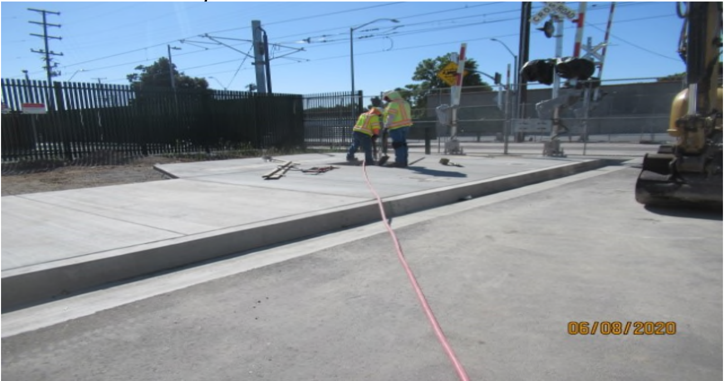
High Street – Select Electric at High St. preparing street light foundation controller box (looking northeast)
