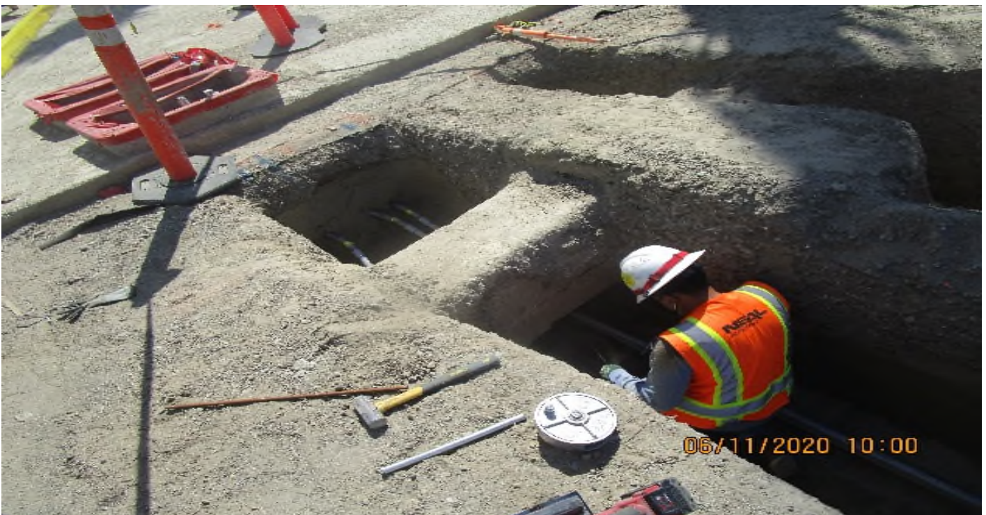
VERNON STATION- Continued rough in underground CCTV & power (JB-38-175D & JB-76-775D) to 18"x18"x8" PB's.
