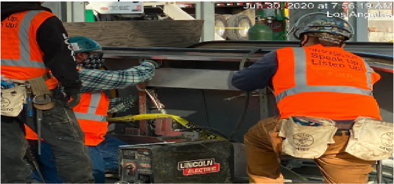
LEIMERT PARK STATION – Installing handrail backer for Escalator 1 at the main entrance landing.
