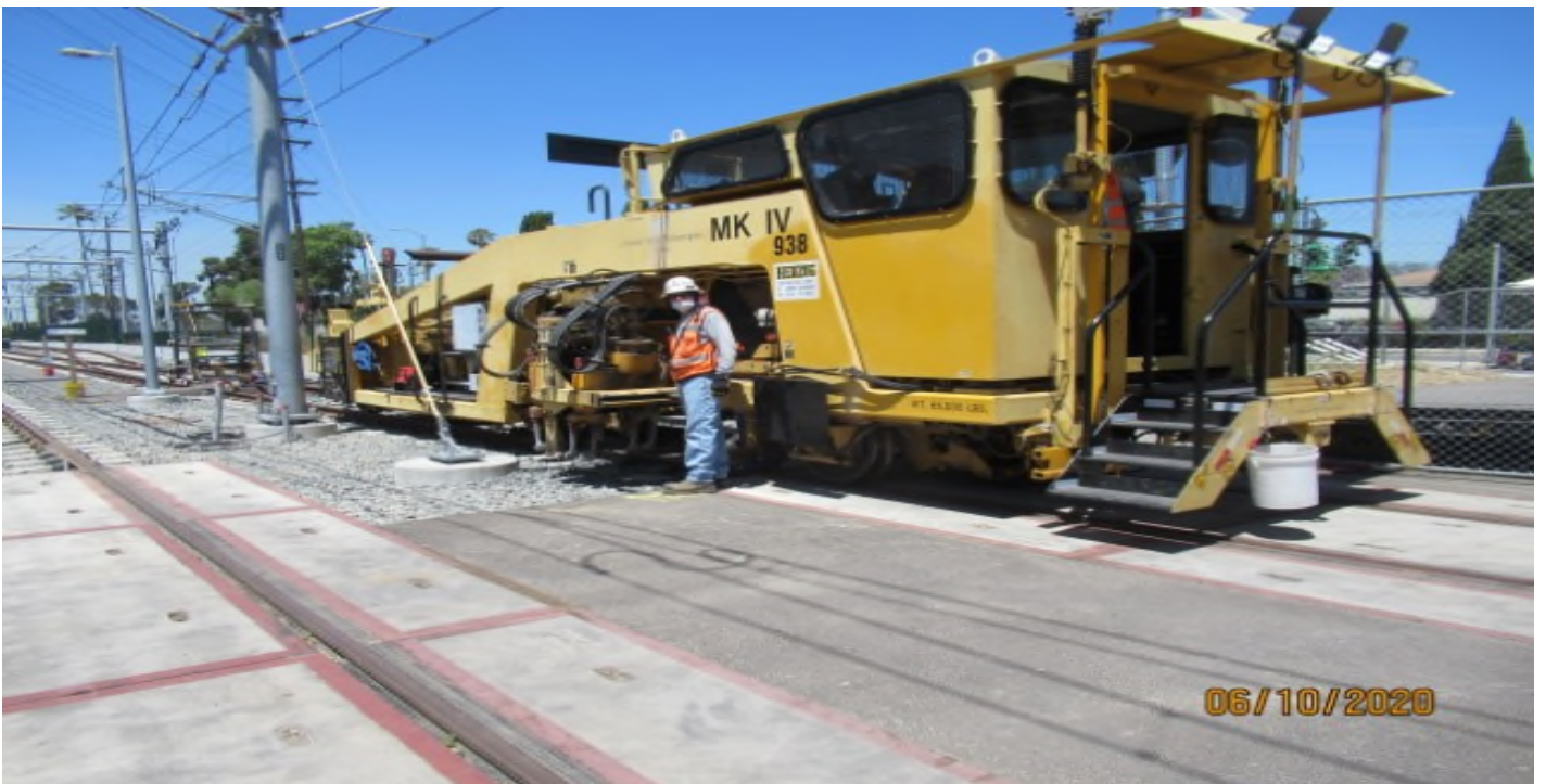
High Street – HCC’s Mark IV tamper at High St. on SB #3 (looking south west)
