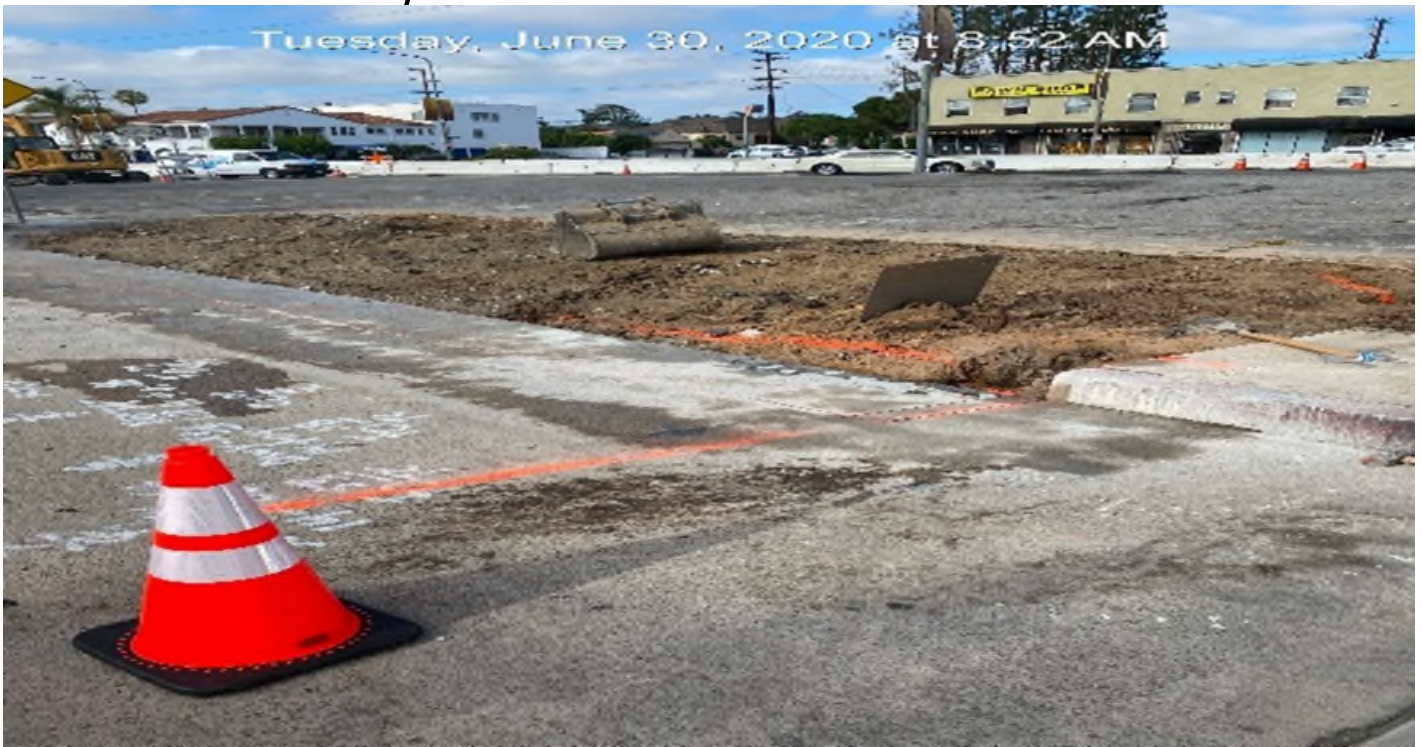
LEIMERT PARK STATION – Excavating/demolishing existing driveway at southbound Leimert Blvd and Crenshaw Blvd.
