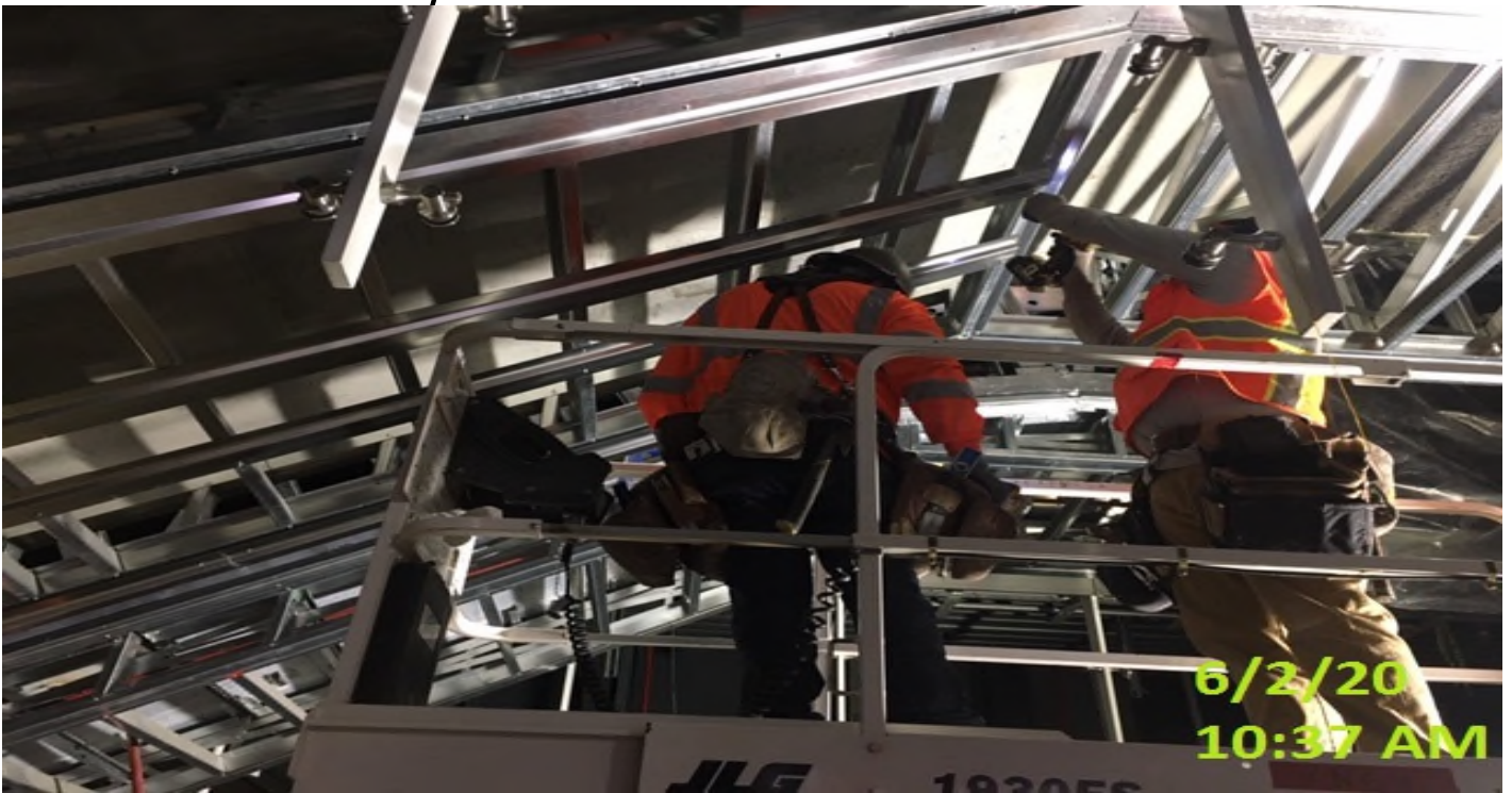
EXPO STATION – Installing stainless steel vertical channels underneath staircase 2 at the platform level.
