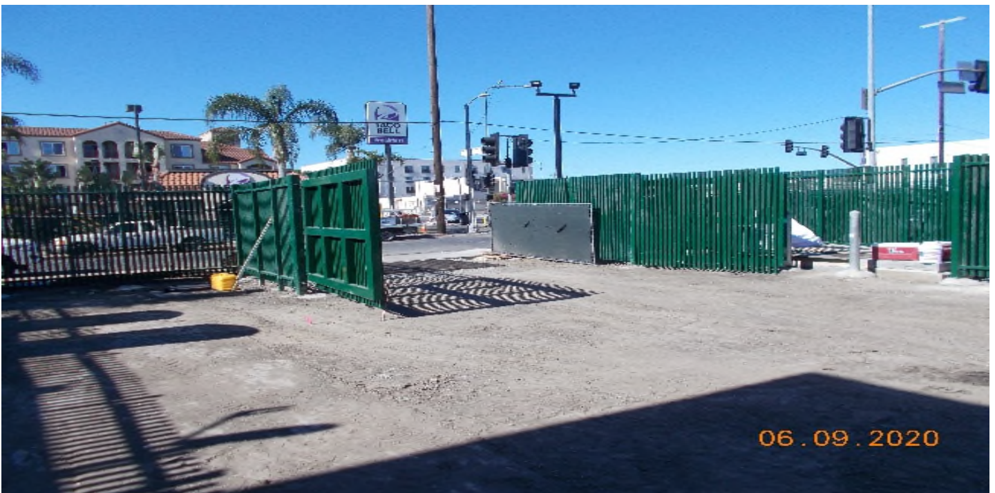
PARK MESA – Completed swing gate installation at the entrance of TPSS#7 on 60th St & Crenshaw Blvd.
