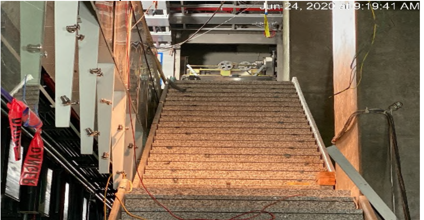
LEIMERT PARK STATION – Continue installing granite riser and threads for staircase #3 from concourse to platform level.
