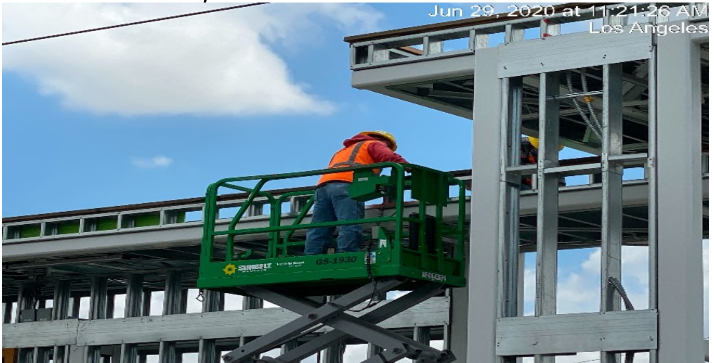
Hyde Park Station – Forming roof for the north canopy structure at the platform.
