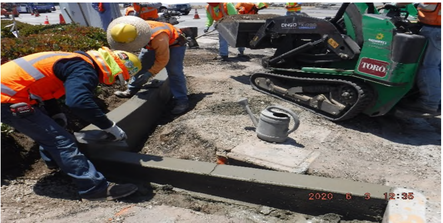
AVIATION/CENTURY- STA 55+00 at Aviation Blvd , 104th St looking south – sidewalk PCC pour SE corner of the intersection.
