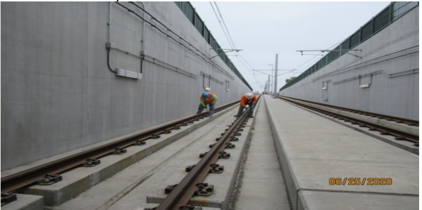
UG1- WSCC adjusting E-clips on NB #4 track UG1 south portal (looking south) Rework
