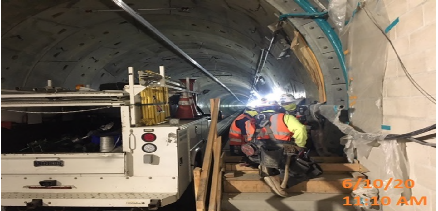
EXPO STATION – Installing embedment at the stair landings of the northbound emergency walkway in the invert level.
