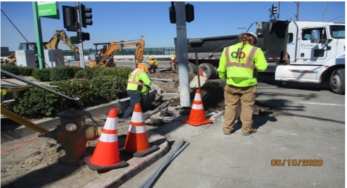
104th Street- Trenching and placing conduit for a future light pole at 104th street.
