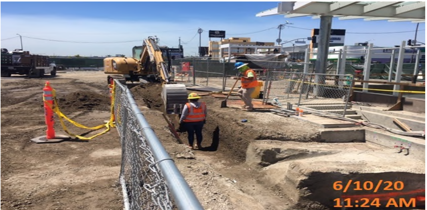
EXPO STATION – Continue excavating/trenching for underground conduit installation for landscape lighting/utilities and irrigation at the plaza level.
