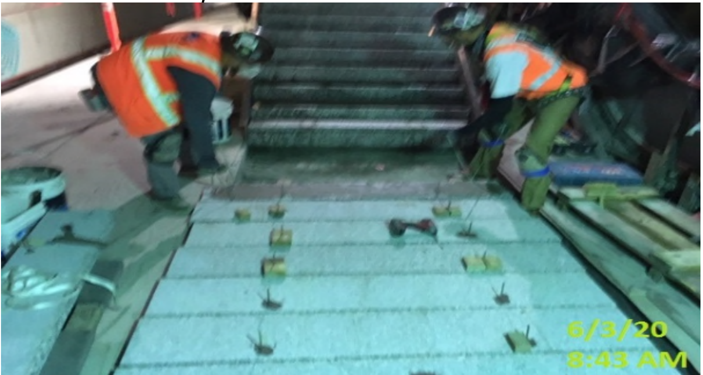
LEIMERT PARK STATION – Continue granite tread and riser installation for staircase #4 from concourse to platform level.
