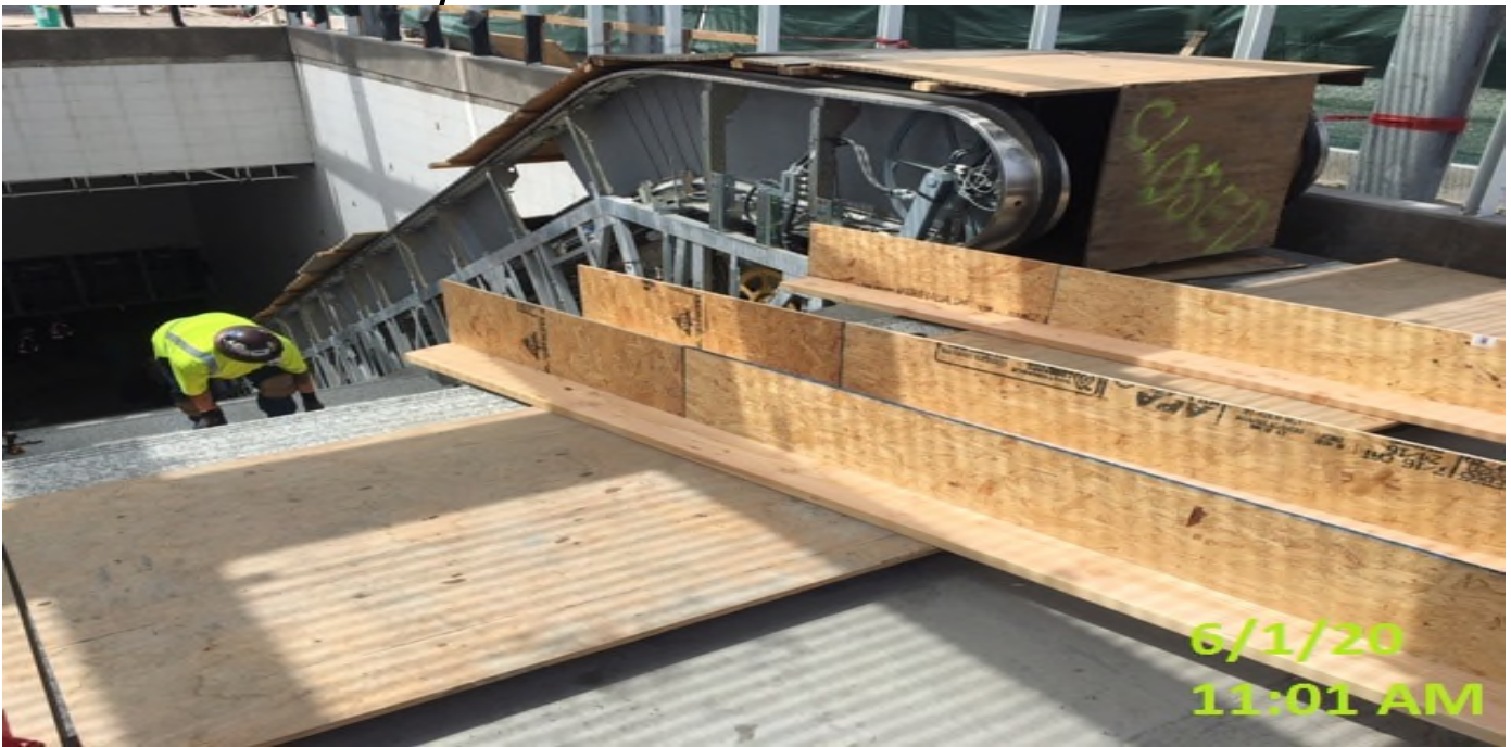
EXPO STATION- Carrera Marble wrapping completed sections of main staircase in plywood.
