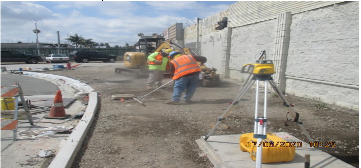
UG3 – Grading for sidewalk installation for a section of the Victoria Cul-de-sac radius. 6/17/20
