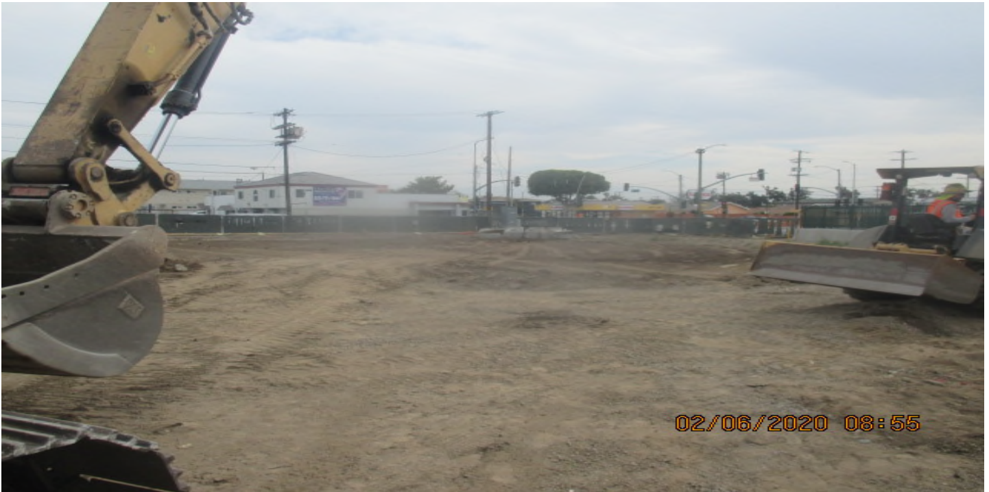
UG3 – Continue excavating/grading the north east section of Victoria Yard for upcoming pavement installation. 6/2/20
