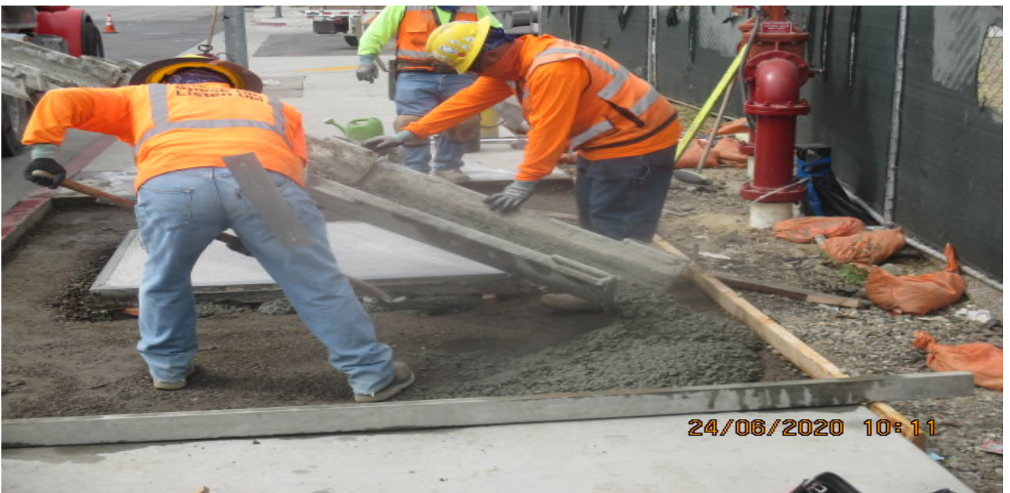
PARK MESA – Placing concrete for new bud pad installation on the southwest corner of 67th St & Crenshaw Blvd. 6/24/20
