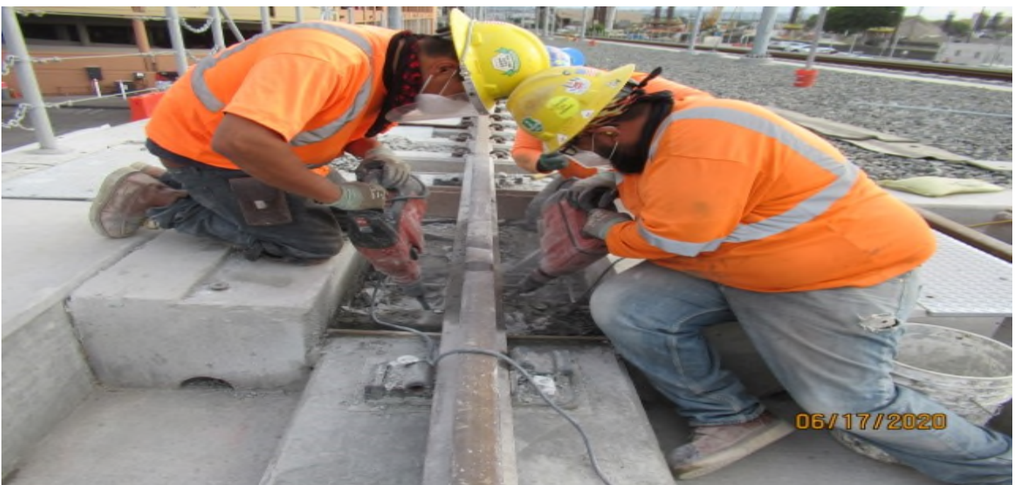
AVIATION/CENTURY- SB #3 track STA 74+60, WSCC concrete demolishing partial plinth left (high) side of curve 7A (looking north) Rework.
