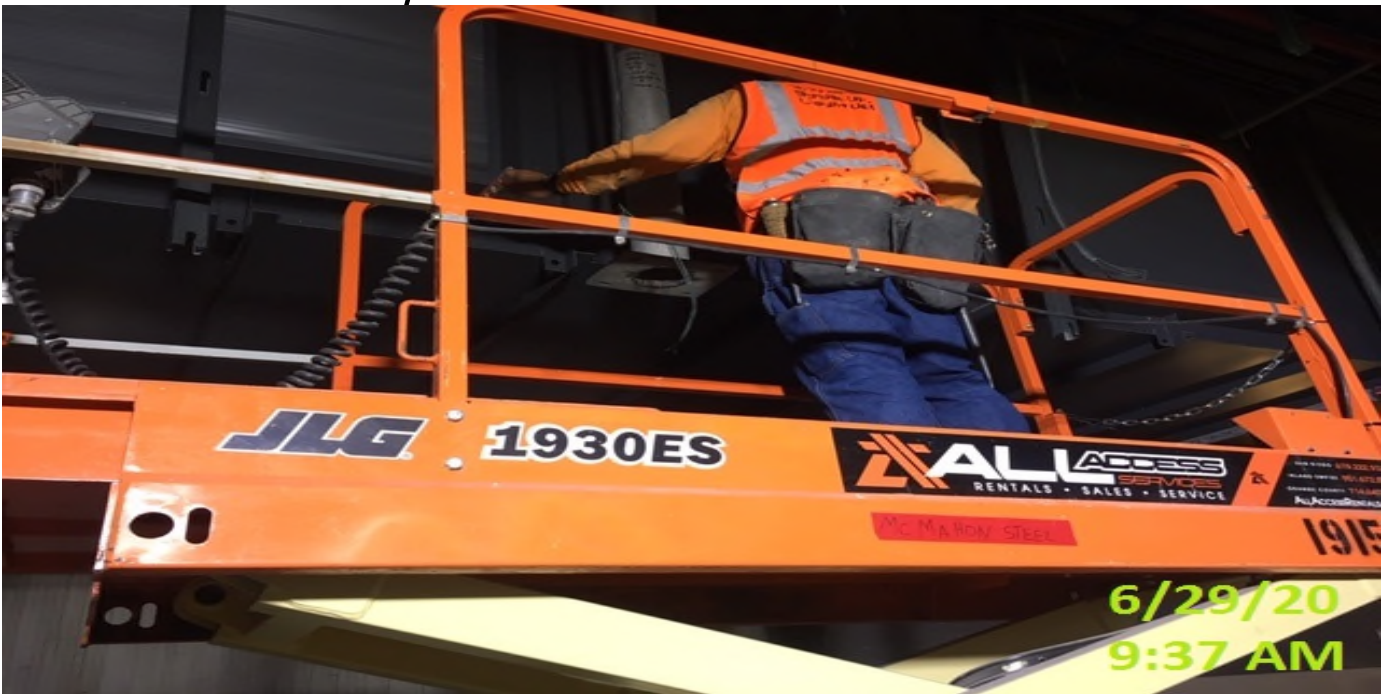
EXPO STATION – Continue welding southbound edge light support poles along the platform level.
