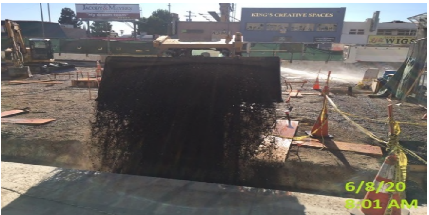
MLK - Backfilling the encased 12” HDPE drainage pipe line at the plaza level.
