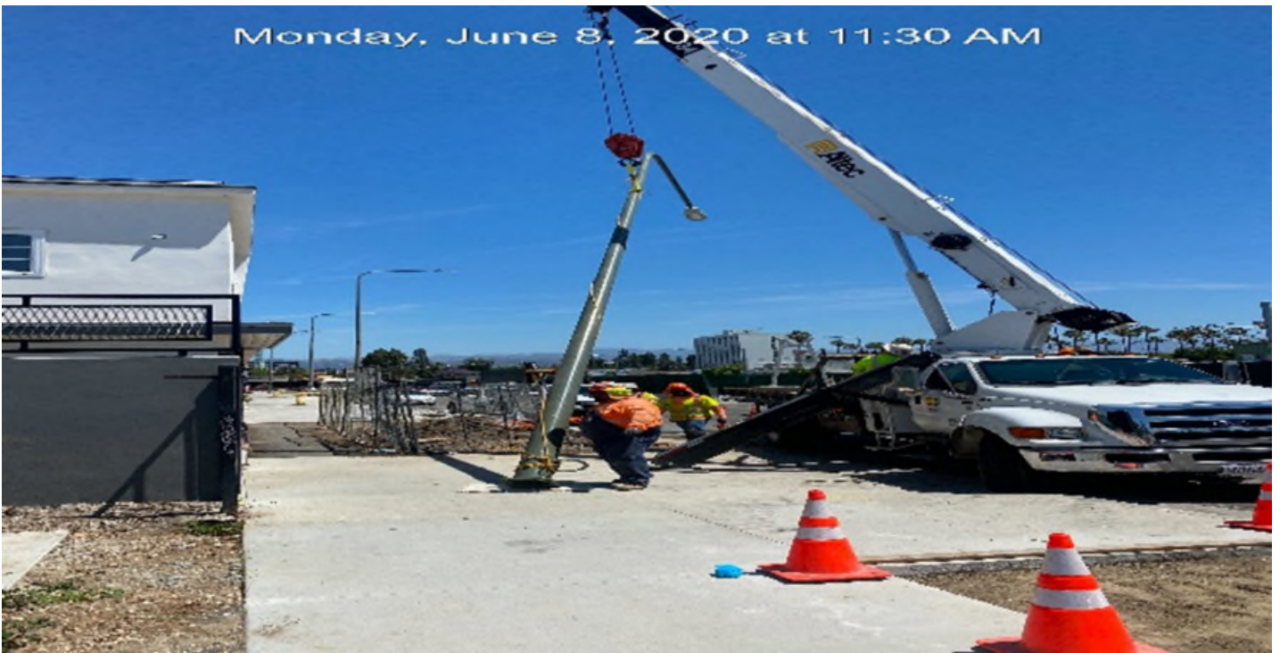
LEIMERT PARK STATION – Installing street light pole on southbound Crenshaw Blvd between 48th St and Brynhurst Ave.
