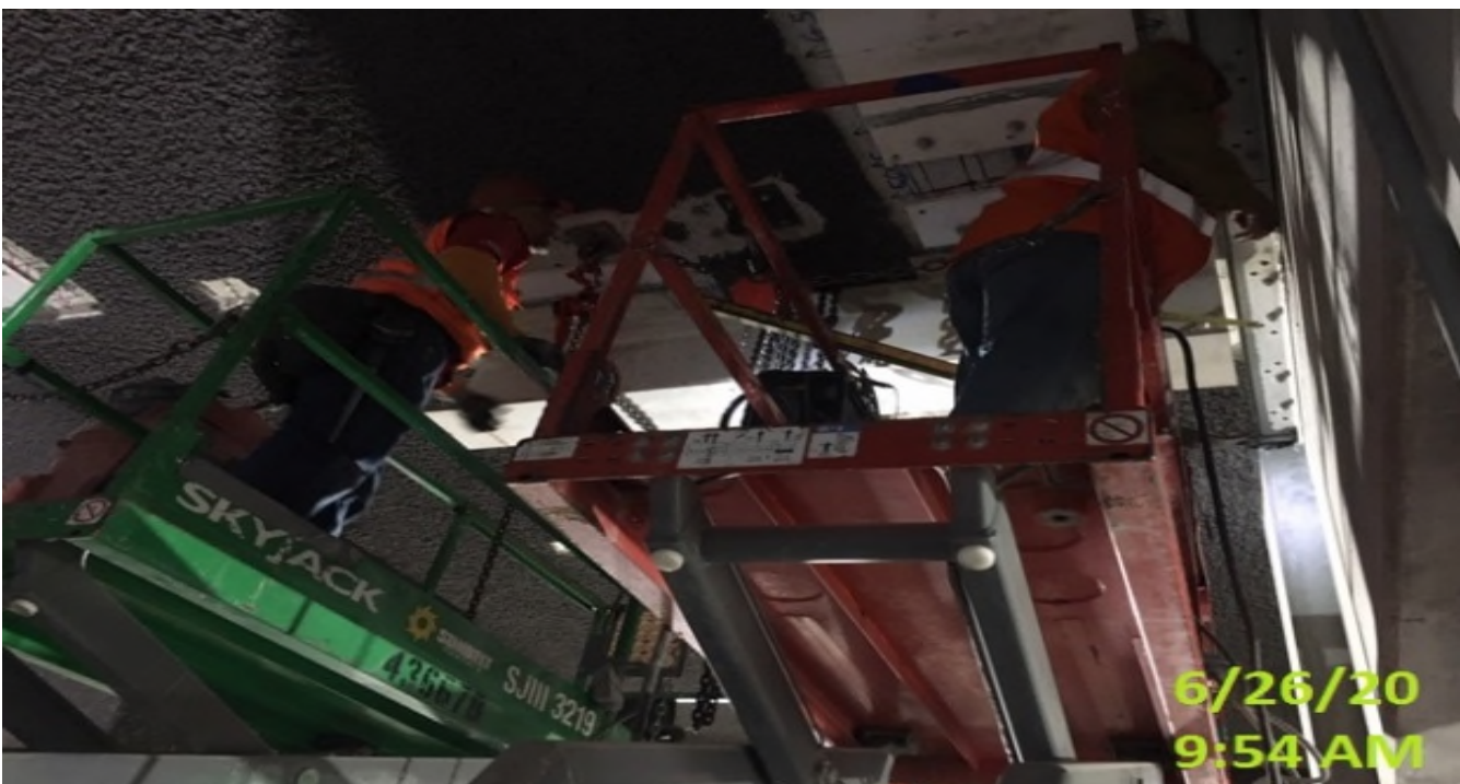
EXPO STATION – Placing and anchoring structural beams to ceiling plates in the North Fan Room of the concourse level.
