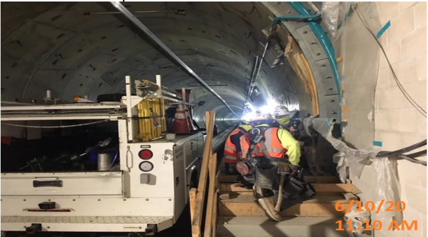
EXPO STATION- WSCC crew installing embed for stair landing at emergency walkway.
