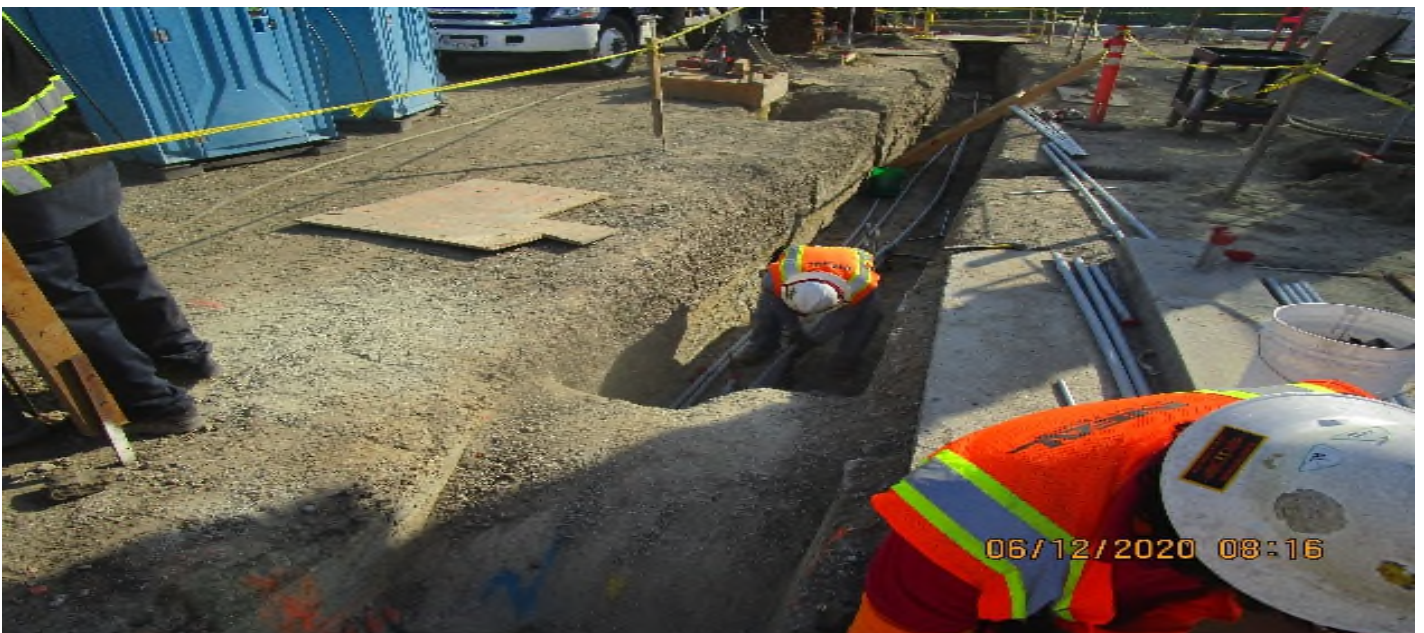
LEIMERT PARK STATION – Continue underground conduit installation for landscape lighting and utilities at the plaza level.
