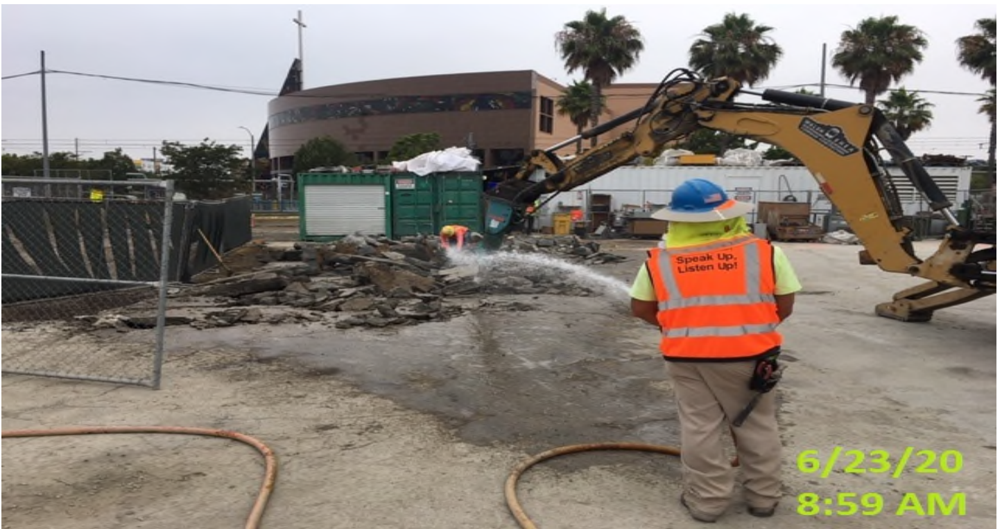
EXPO STATION- WSCC crew demoing and removing concrete slab for park and ride.
