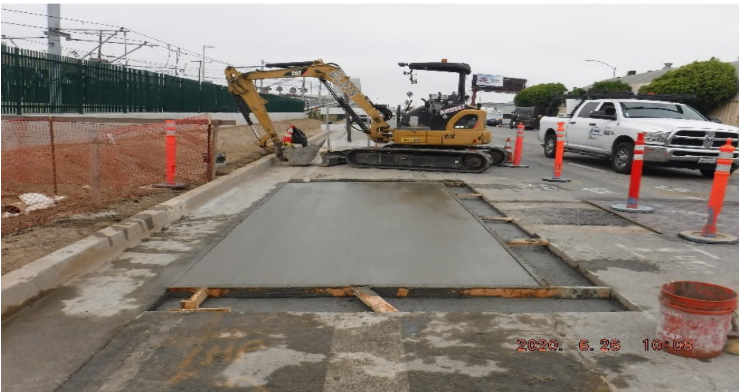
AVIATION/CENTURY- STA 59+00 looking north – Aviation – fresh PCC road surface on top of 8" DWP pipe
