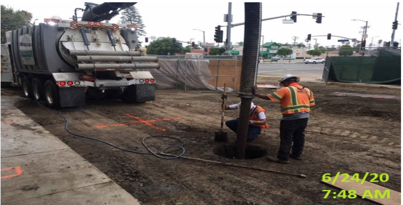
MLK STATION – Potholing for tree wells and underground landscaping conduit installation at the northwest corner of the plaza level.
