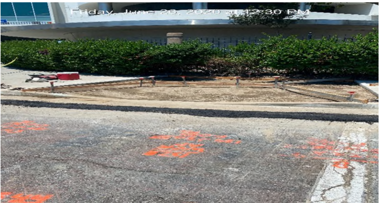
MLK STATION – Continue building formwork and placing concrete for new ADA ramp installation on the northwest corner of MLK Blvd and Crenshaw Blvd.
