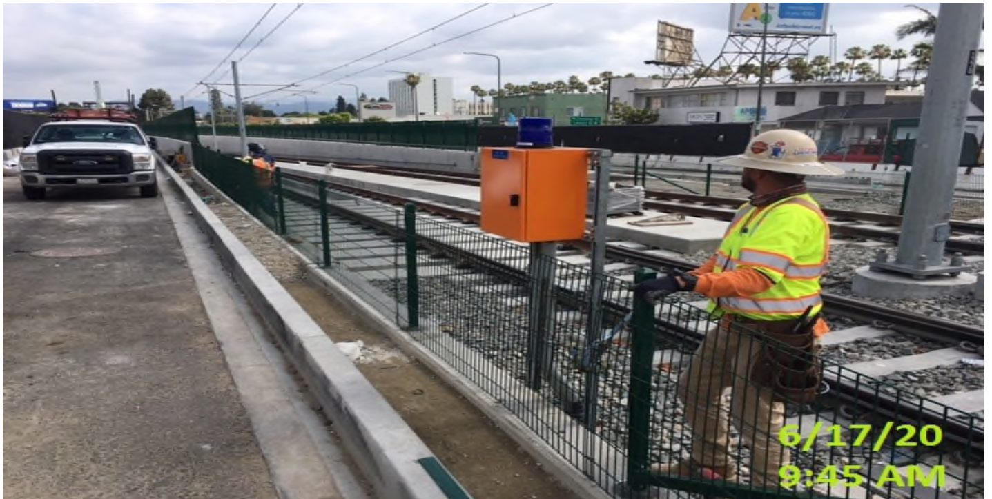
UG4 – Installing fence grill to guardrail posts along both sides of the guideway curb from Sta 317+75 – 322+40.
