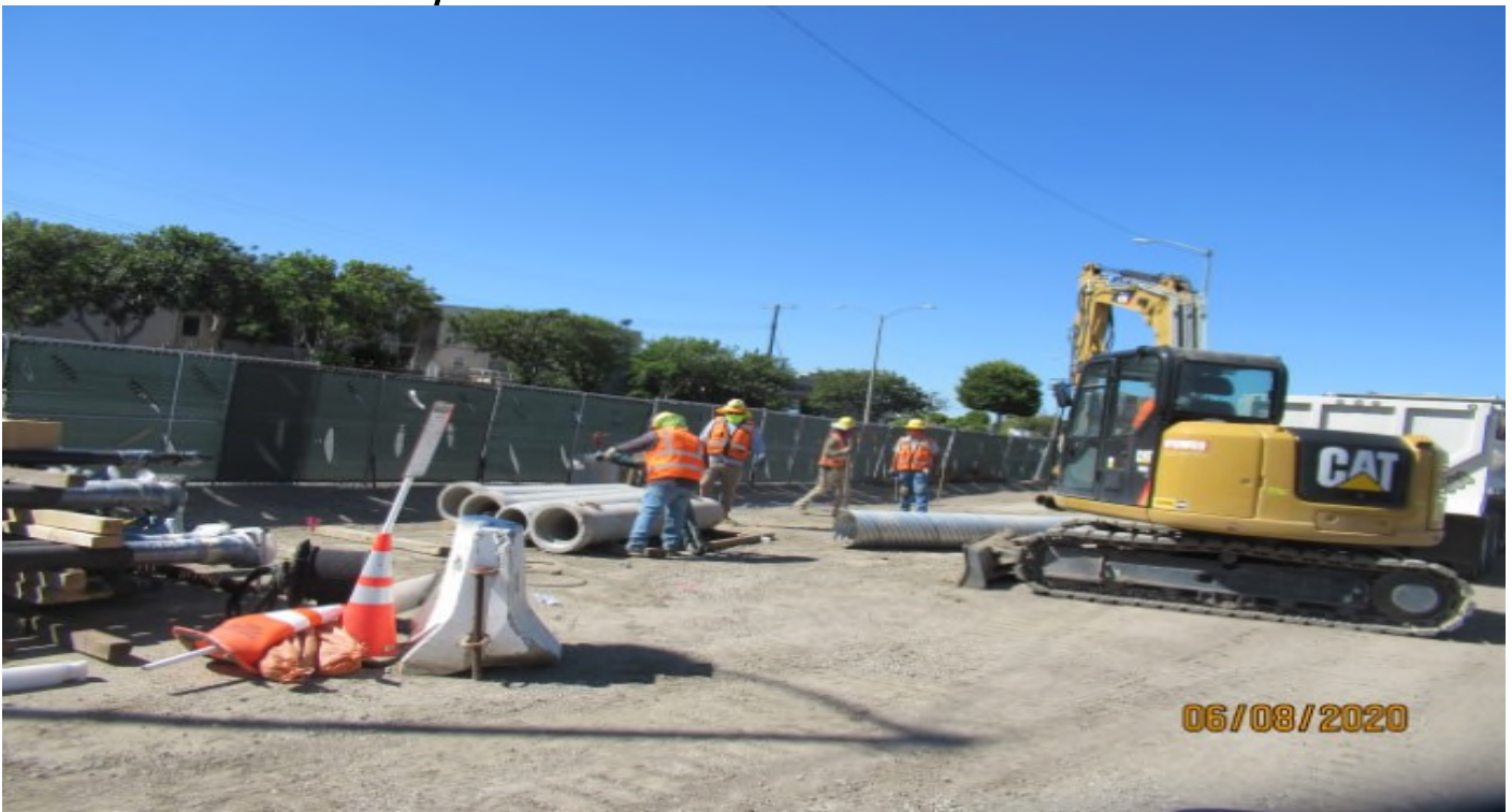
La Brea – WSCC at La Brea pavilion removing materials using excavator (looking southeast)
