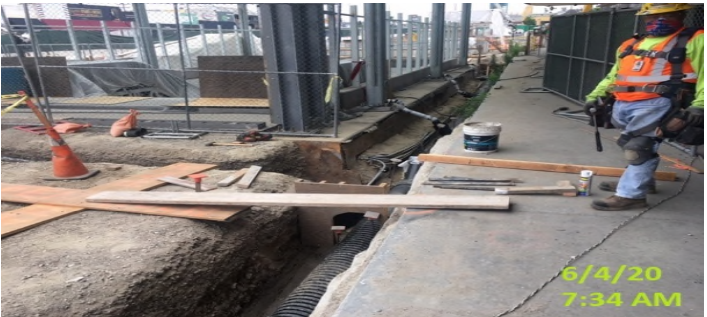
MLK Station - Building and installing bulkheads for slurry encasement of the 12" HDPE drainage pipe at the plaza level.
