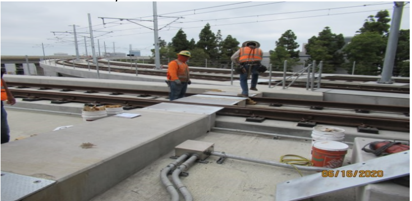
GREENLINE UNDERPASS- WSCC on east leg of Wye, repairing emergency walkway crossings (looking southwest) Rework
