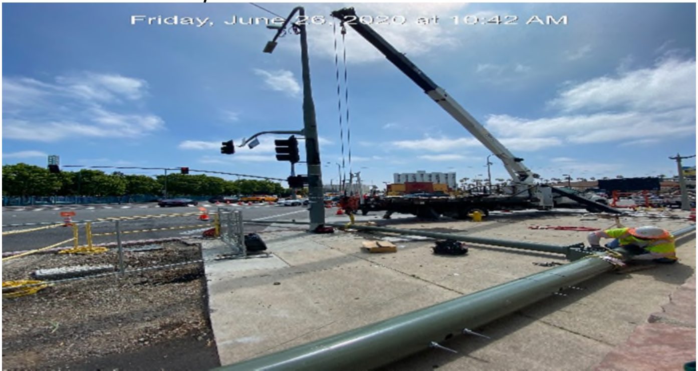
LEIMERT PARK STATION – Installing street light pole on the southwest corner of Vernon Ave and Crenshaw Blvd.
