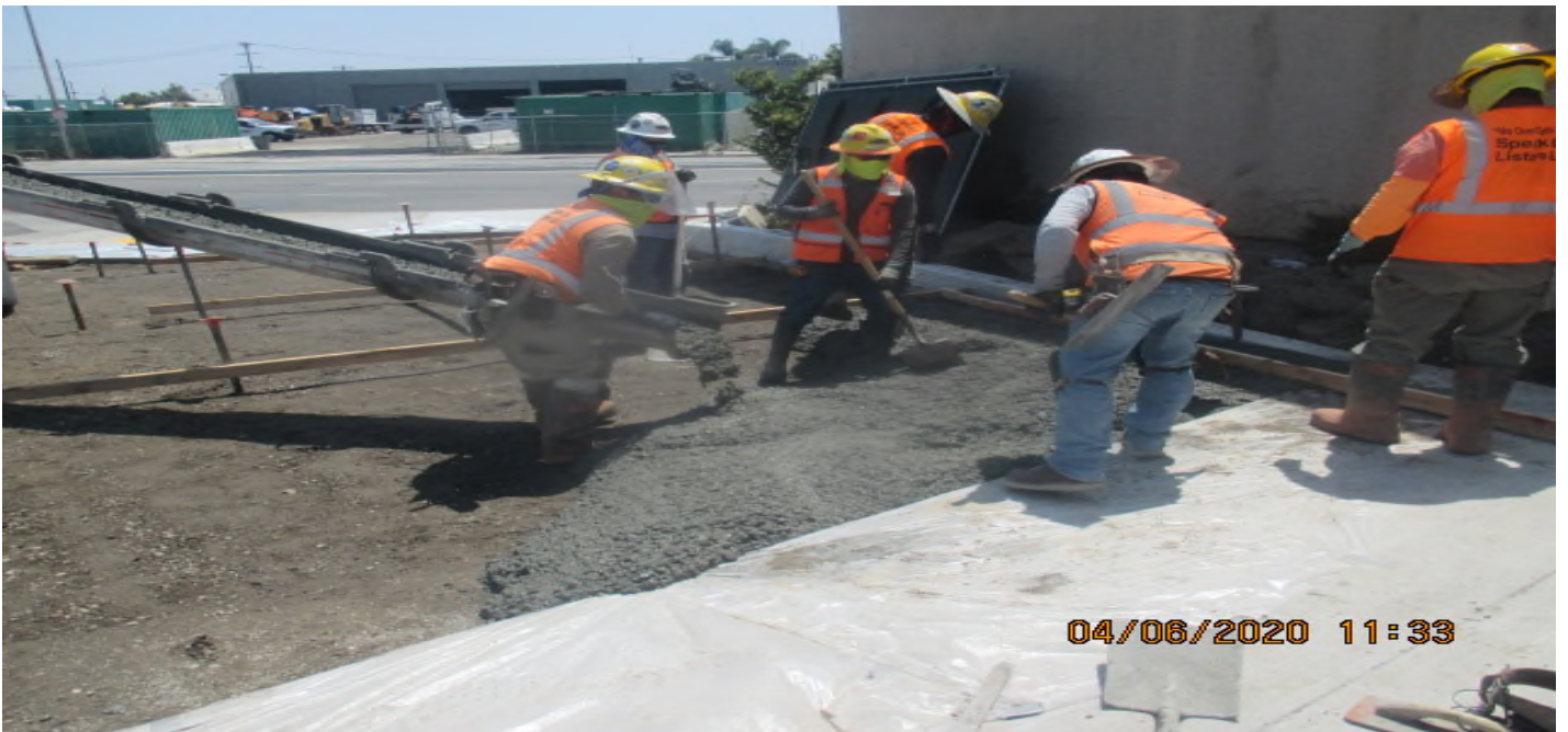
UG3 – Building and installing block-out forms and placing concrete on the southwest corner of “New Road” and Crenshaw Blvd.
