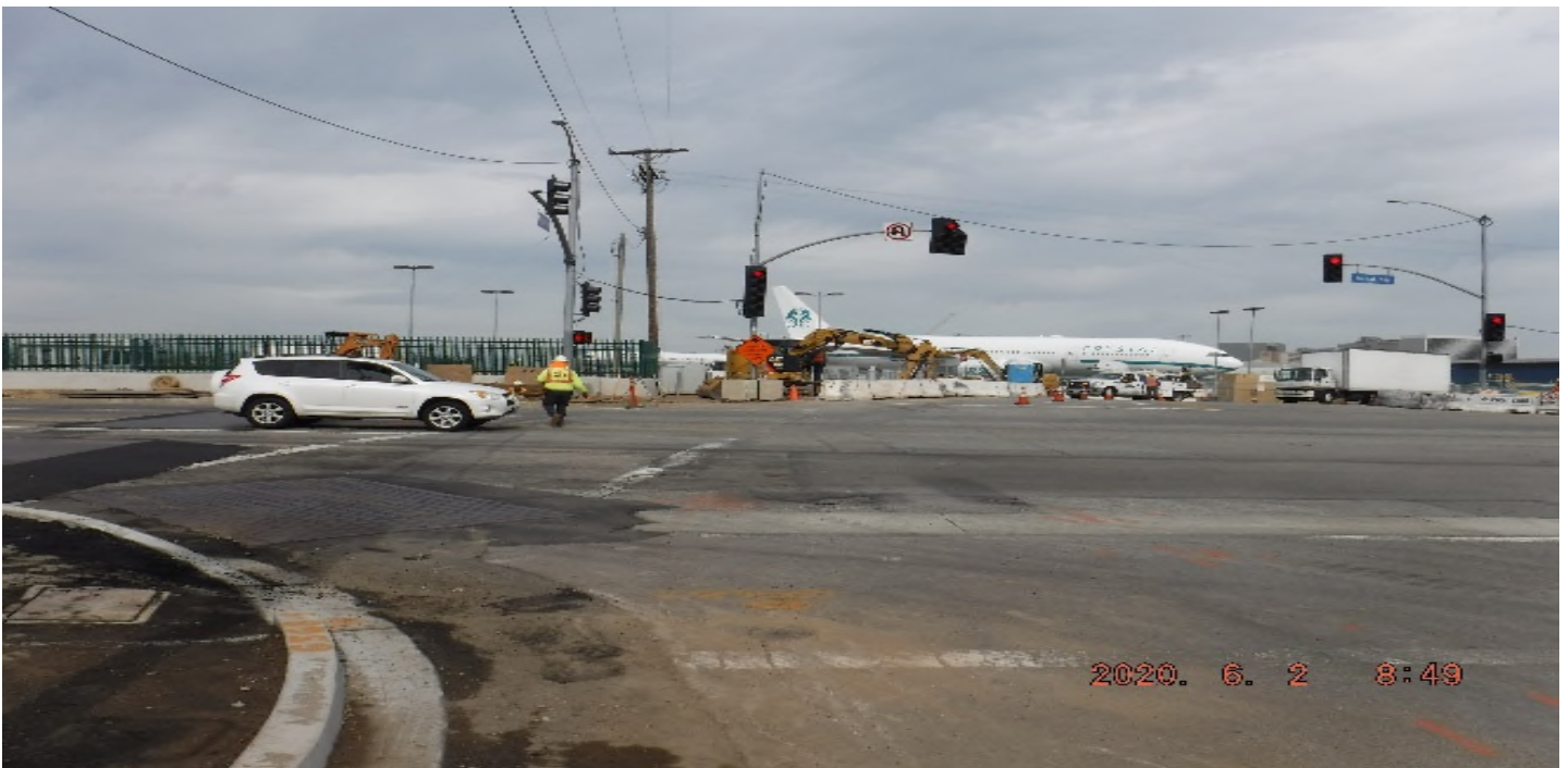
104th Street- STA 55+00 at 104th St looking west – grading work mobilization SW corner (across Aviation/background)
