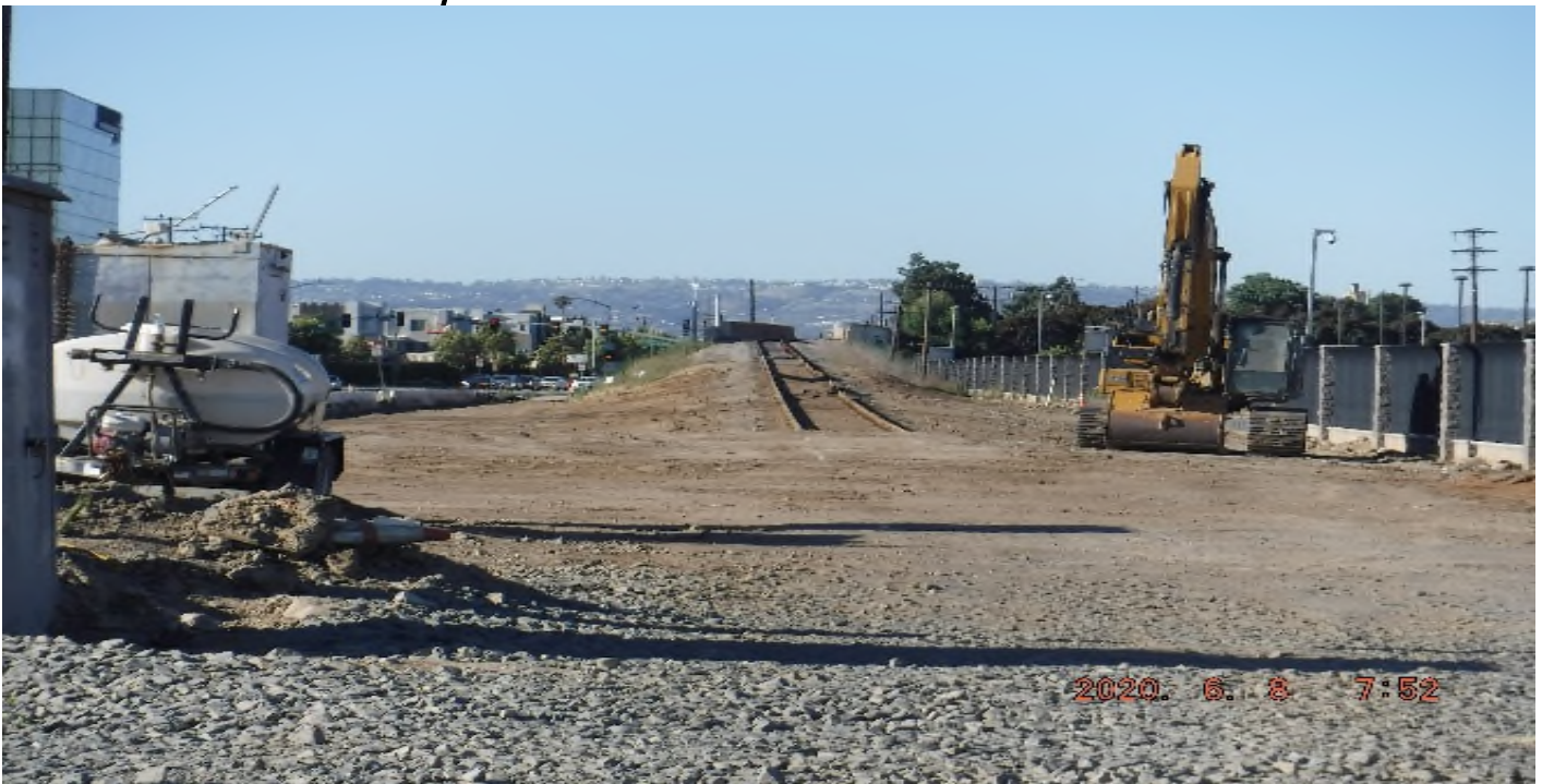
AVIATION/CENTURY- south of 124th St looking south – dirt stockpile removal from BNSF R/W and reclaim the site – on hold
