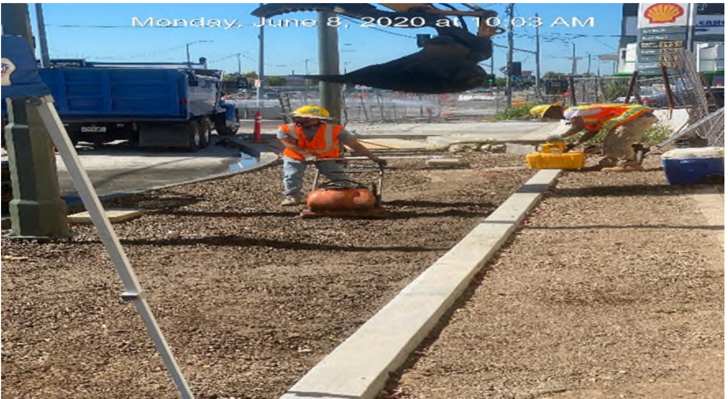
EXPO STATION – Backfilling and fine grading sidewalk on southbound Crenshaw Blvd between Exposition Blvd and Obama Blvd.
