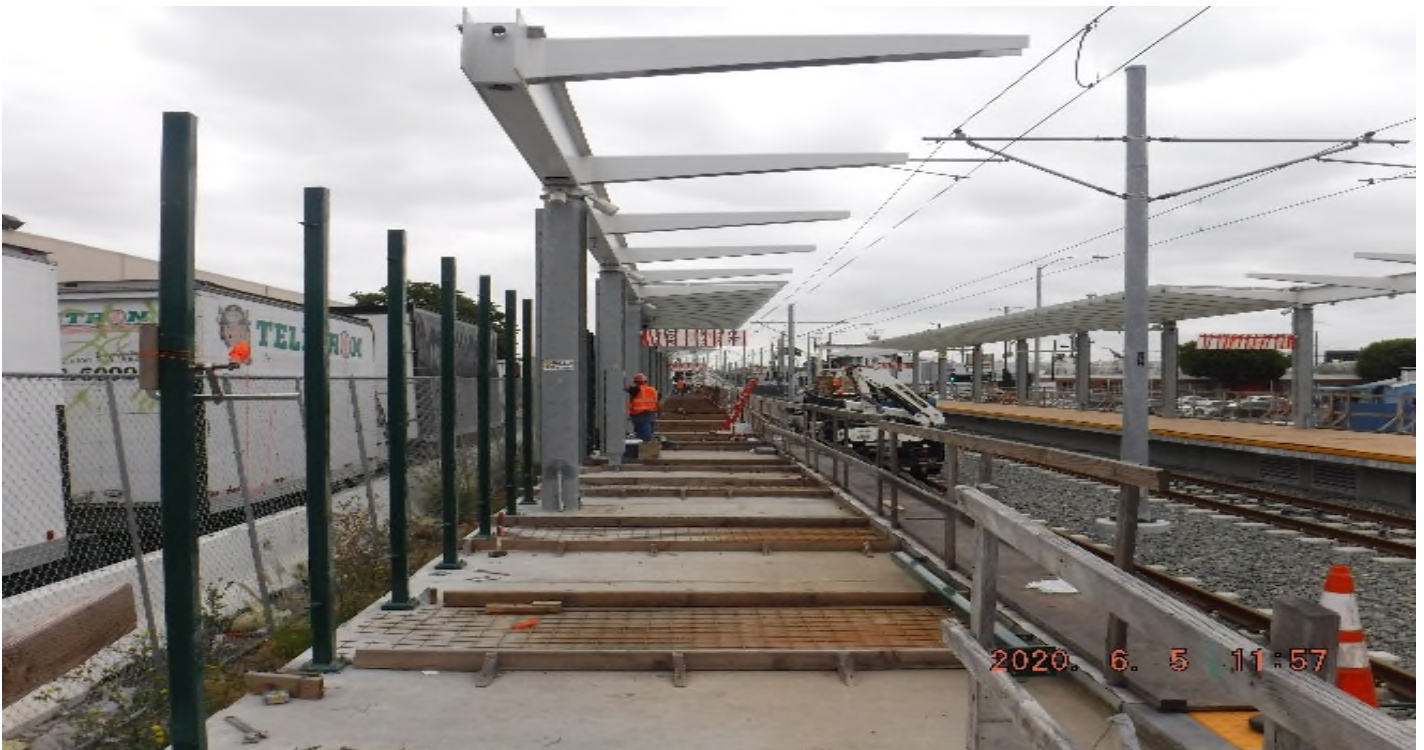
Hindry Station – STA 131+00 TK#3/SB looking north – Hindry Station install the 8' fence posts along the backside of the platform
