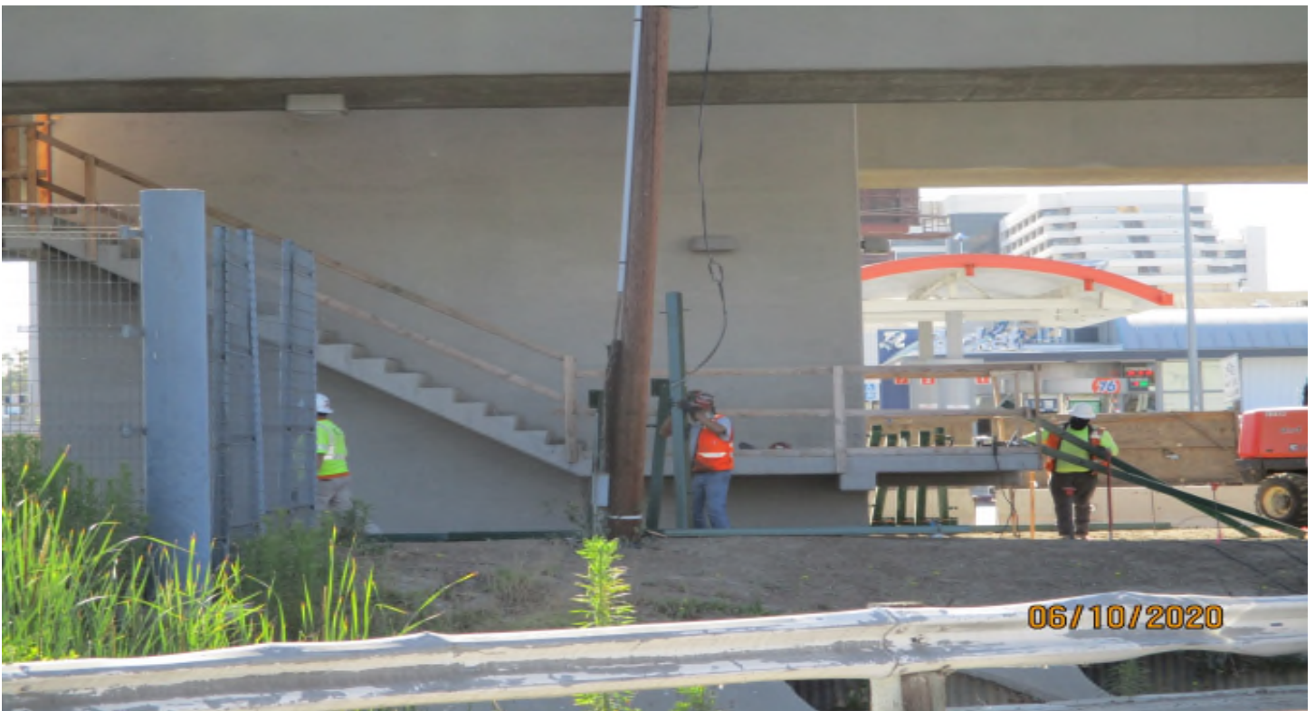
AVIATION/CENTURY- Welding and setting fence posts at the Aviation Station south stairway.
