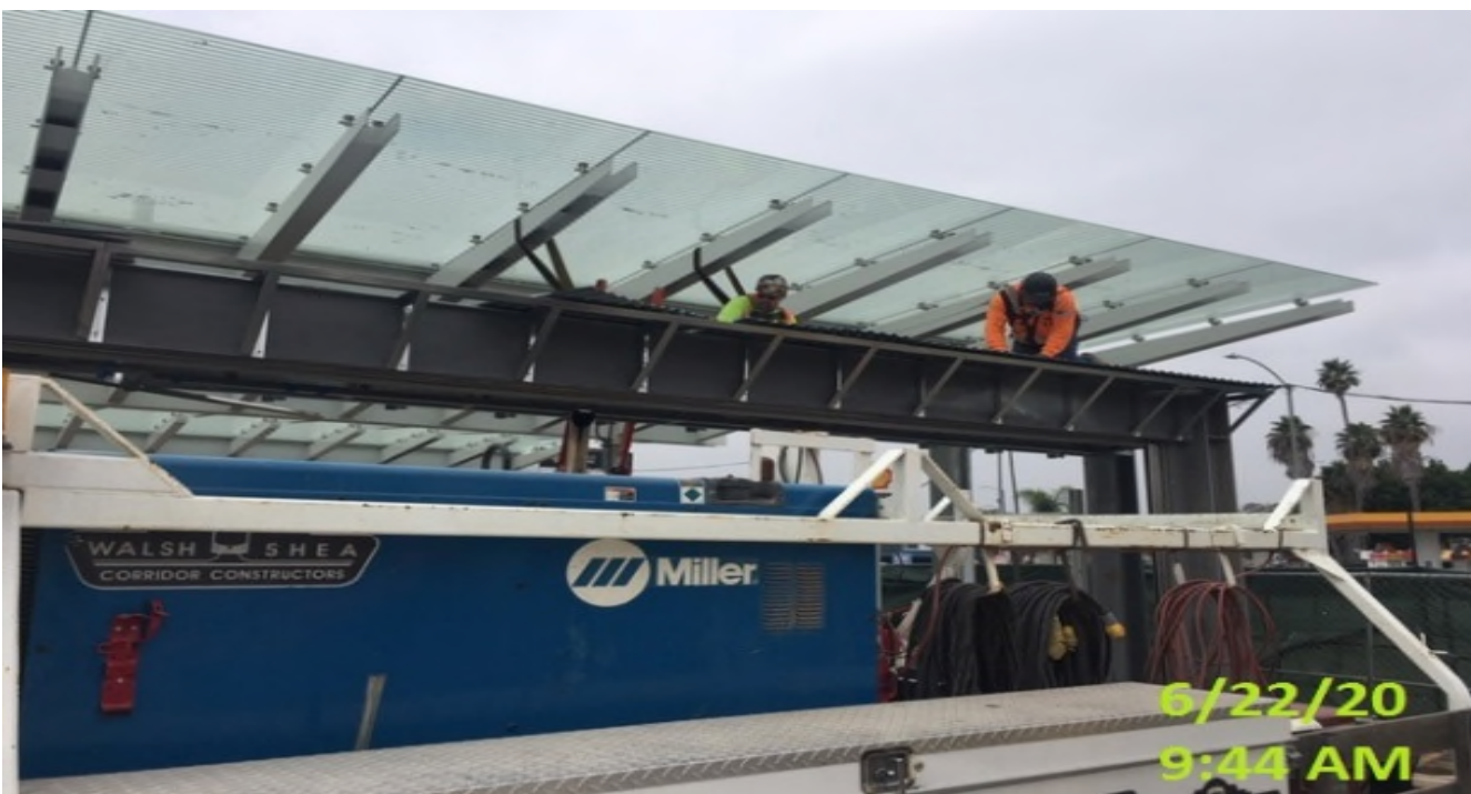
EXPO STATION – Installing roofing deck to the main entrance canopy structure at the plaza.
