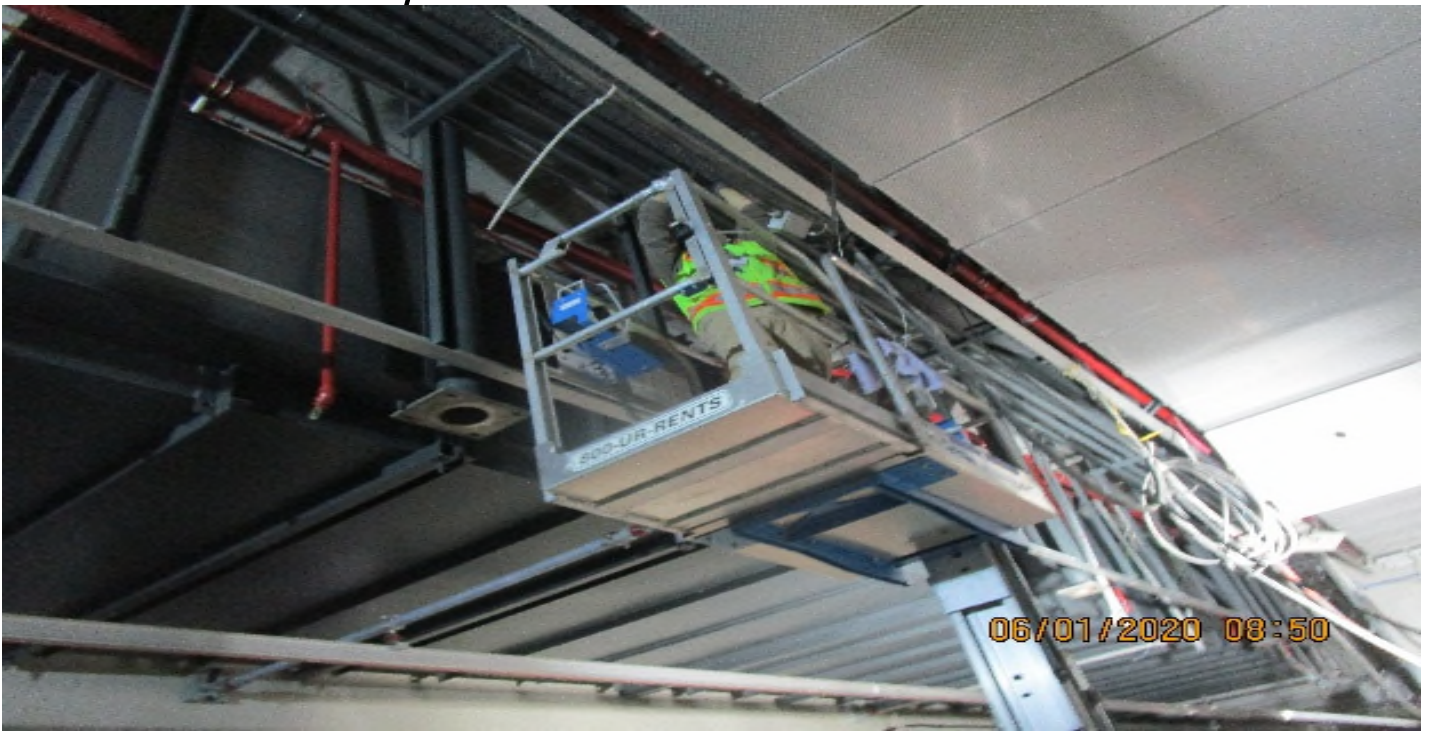
VERNON STATION- GL's 5.5,B.5, Continued piping 2" GRC fire alarm between pull boxes (punch list)
