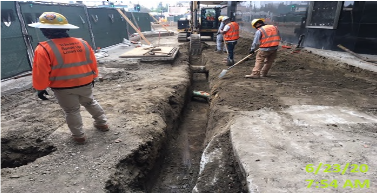
MLK STATION – Excavating/trenching for underground landscaping conduit installation at the west side of the plaza level.
