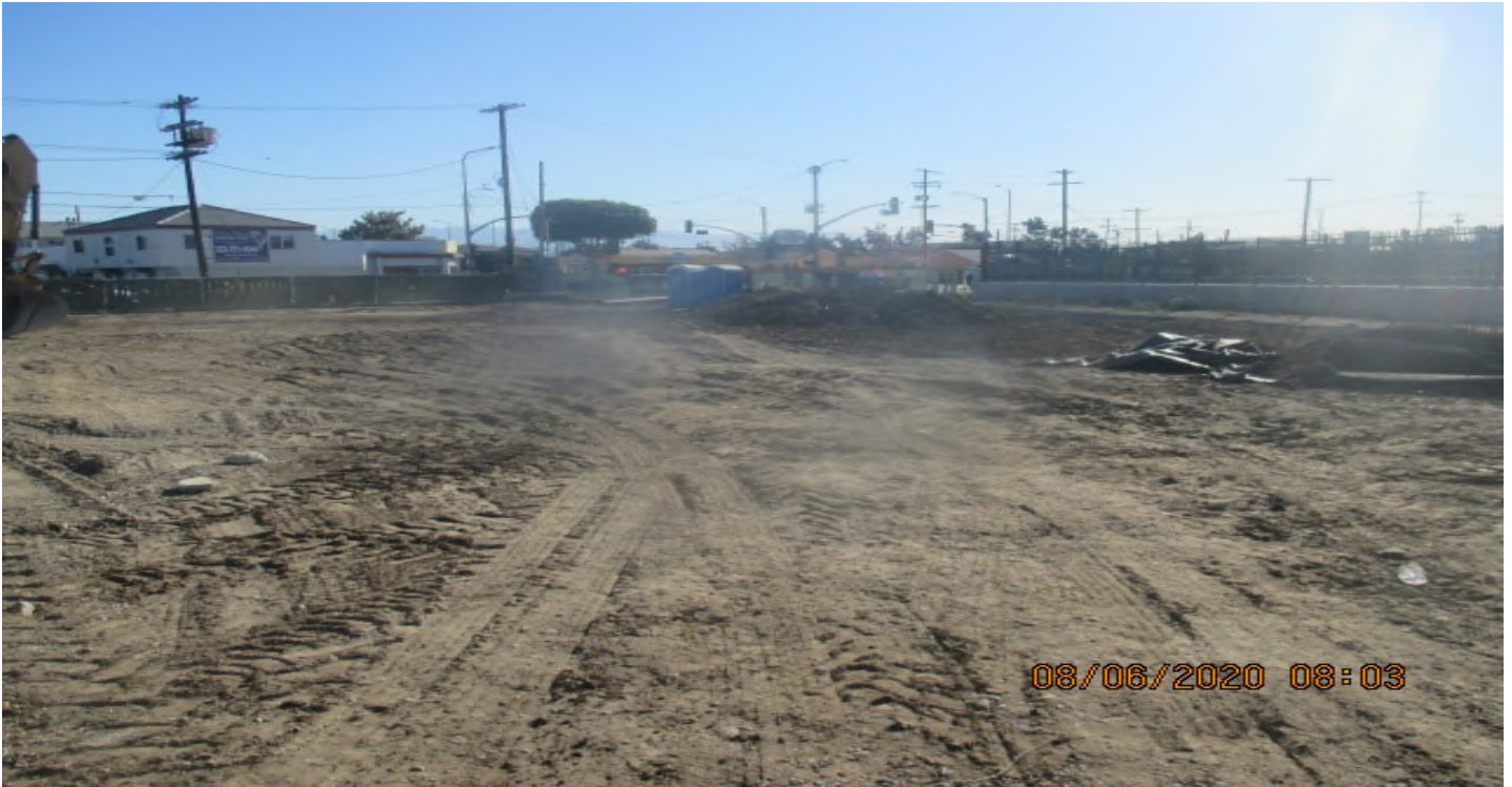
UG3 – Continue grading the north east section of Victoria Yard for upcoming pavement installation.
