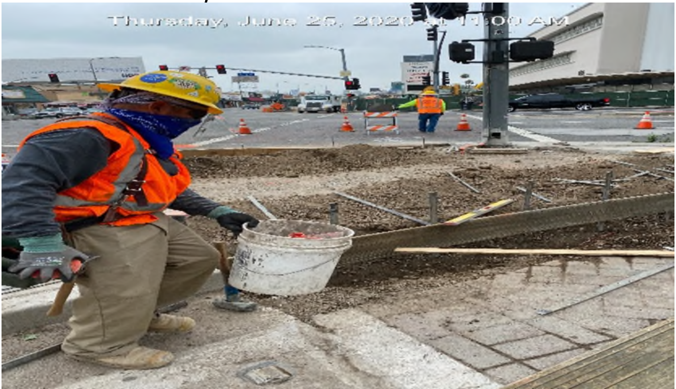
MLK STATION – Building formwork for new ADA ramp and curb/gutter installation on the west median corner of MLK Blvd and Crenshaw Blvd.
