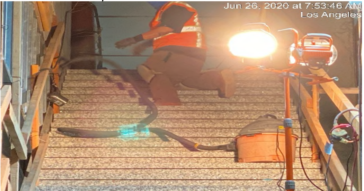
LEIMERT PARK STATION – Continue installing granite riser and threads for staircase #3 from concourse to platform level.
