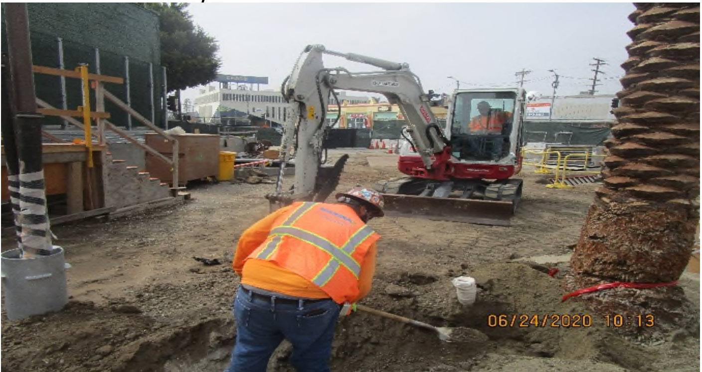
LEIMERT PARK STATION – Continue excavating/trenching for irrigation installation at the plaza level.
