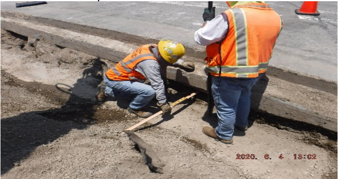
AVIATION/CENTURY- STA 55+00 at Aviation Blvd/104th St looking west – T&M work to expose DWP duct bank – survey.
