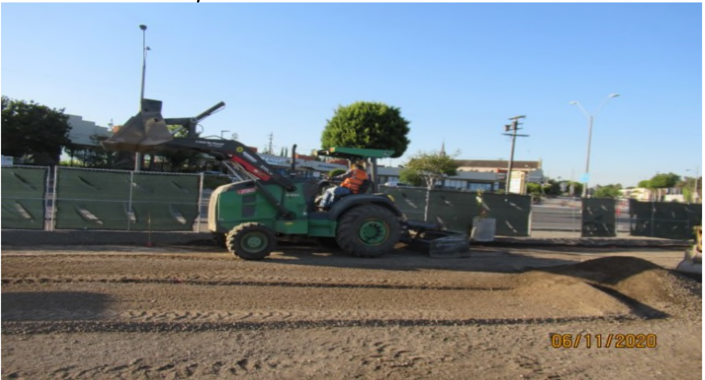
La Brea – WSCC final grading in La Brea parking lot (looking east)
