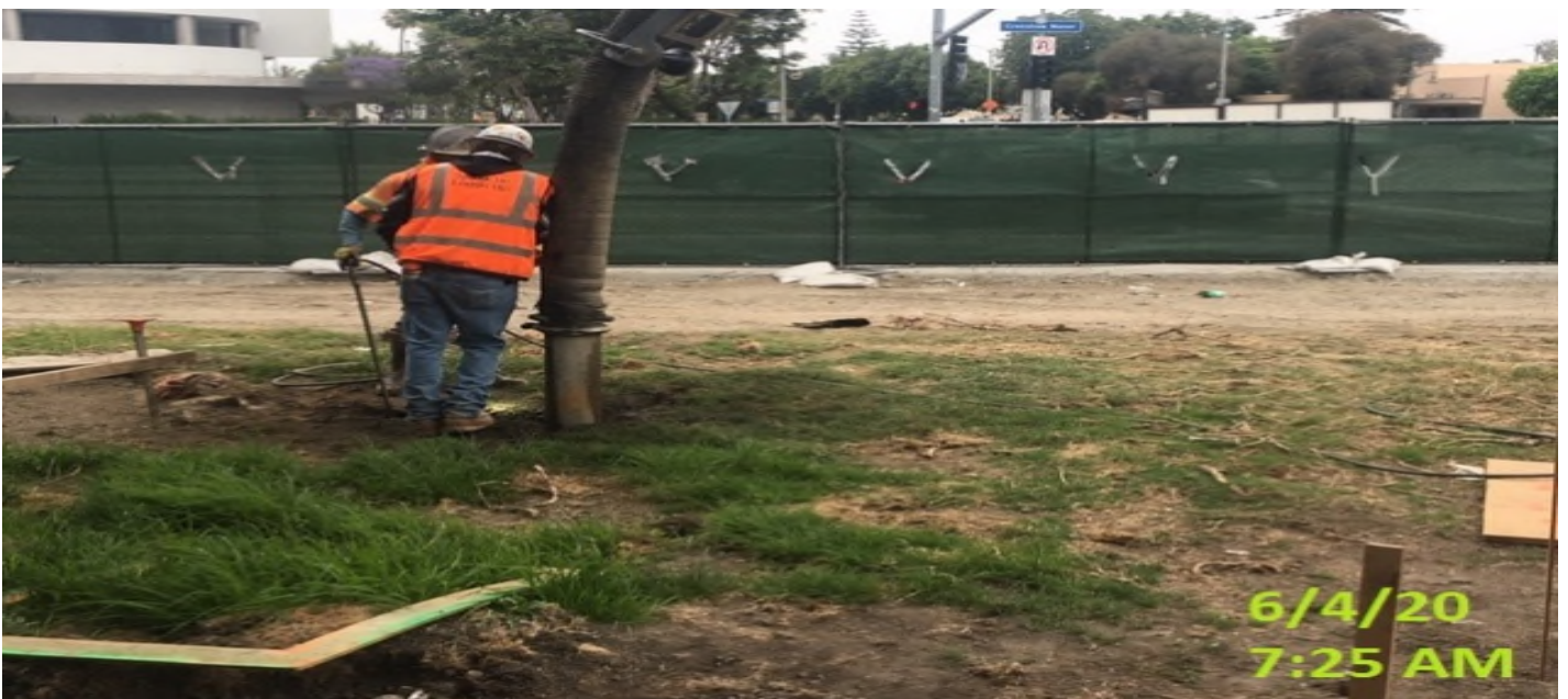
MLK Station - MLK – Continue potholing for the installation of light pole foundations and tree wells at the plaza level.
