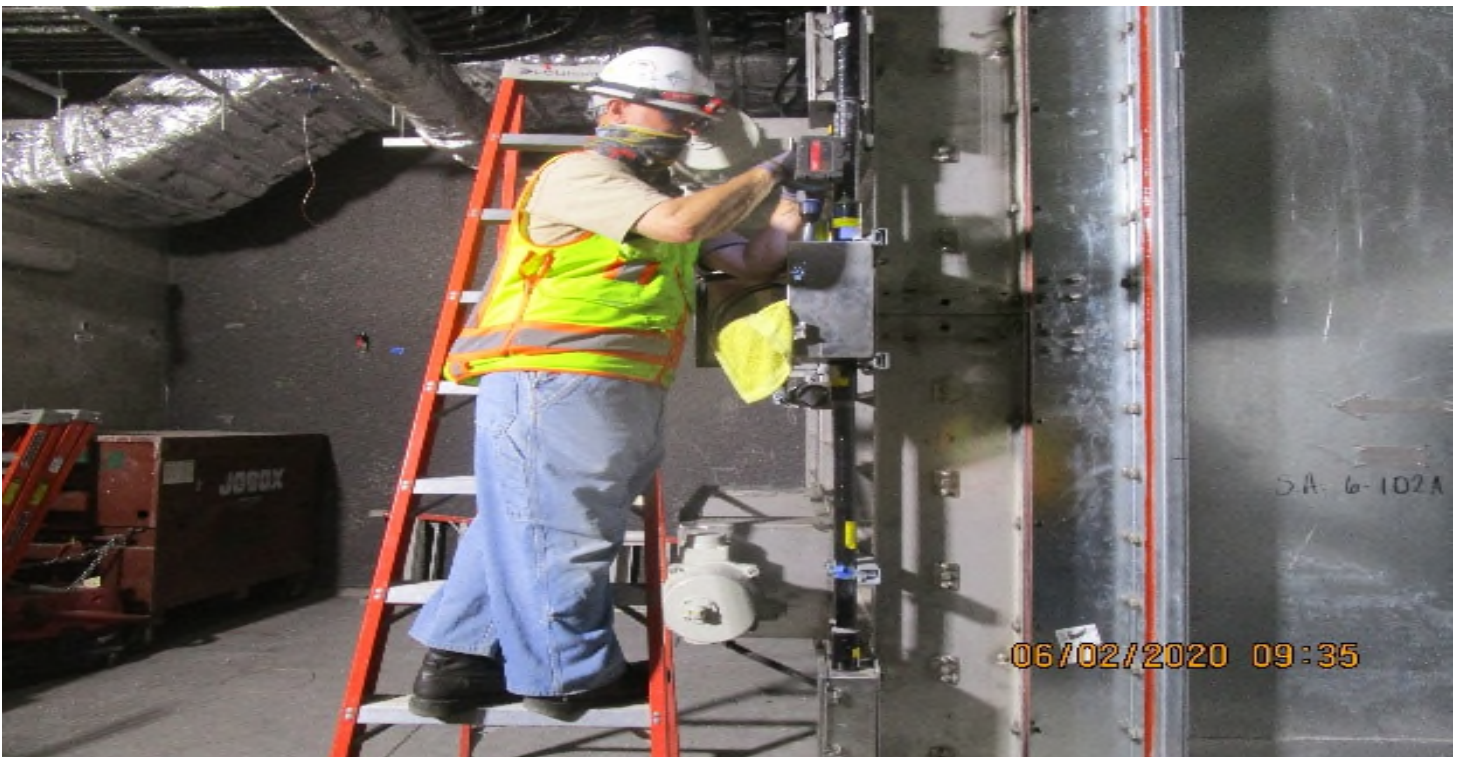
VERNON STATION- Emergency fan room (N) C126, BD-6-102 & TD-6-102 begin installing drains & breathers at Nema4X JB's.
