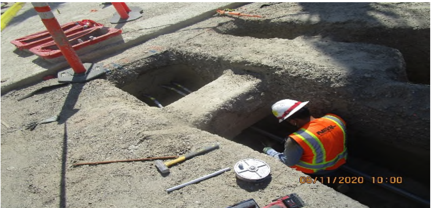
LEIMERT PARK STATION – Continue underground conduit installation for landscape lighting and utilities at the plaza level.
