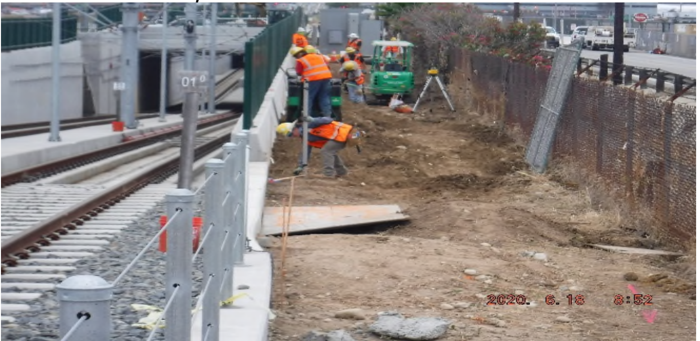
AVIATION/CENTURY- STA 60+50 at Aviation Blvd, 104th St looking south – grading work next to UG1’s left wall toward RW60L.
