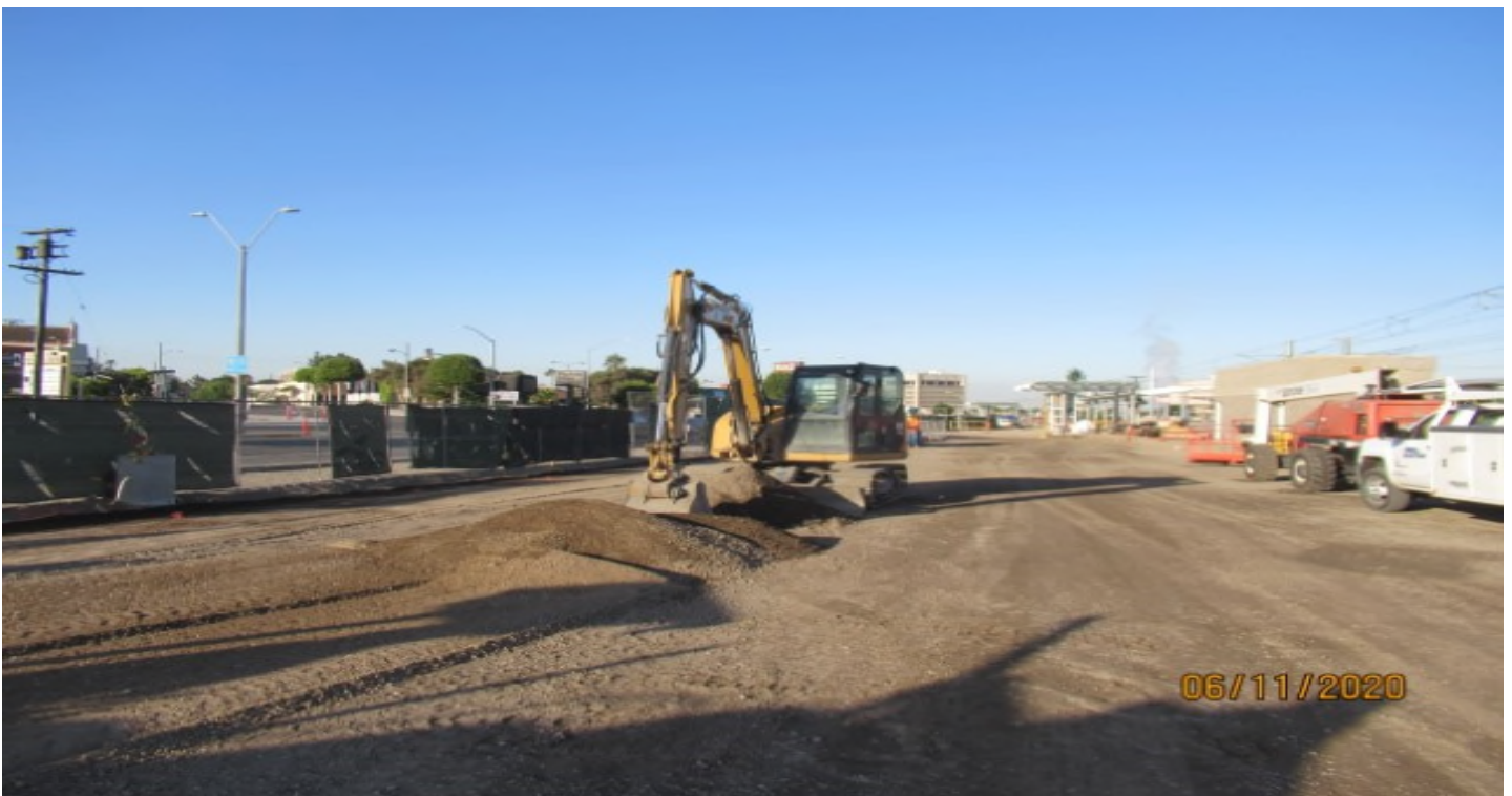
La Brea – La Brea parking lot WSCC final grading CMB (looking south)
