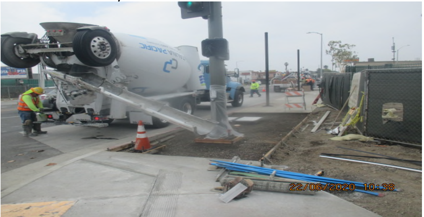
PARK MESA – Placing concrete for new sidewalk panel installation on the southwest corner of 67th St & Crenshaw Blvd. 6/22/20
