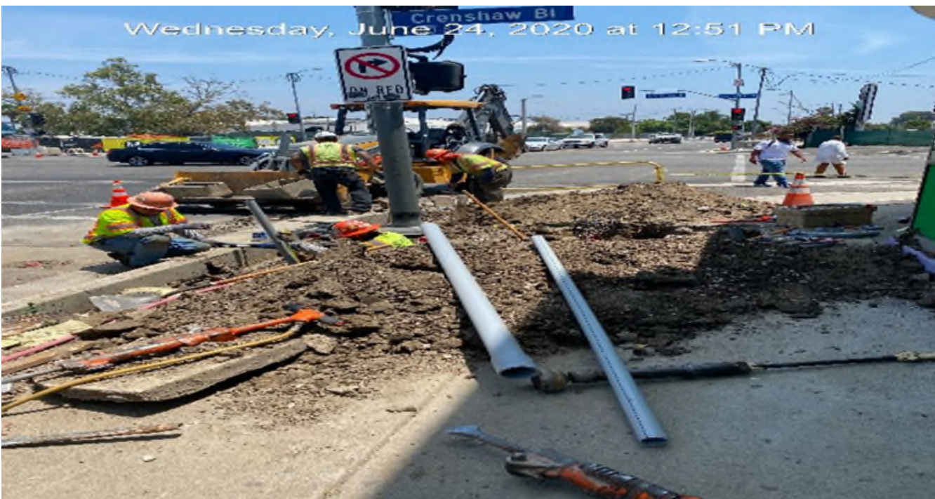
EXPO STATION – Continue installing conduit to supply power for the street light pole on the southwest corner of Obama Blvd and Crenshaw Blvd.
