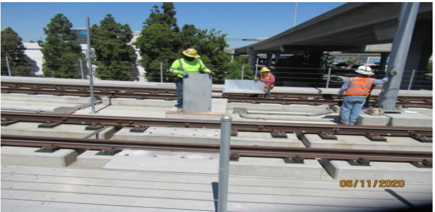
GREENLINE UNDERPASS- WSCC at west leg of GL Wye, installing repaired emergency walkway plates
