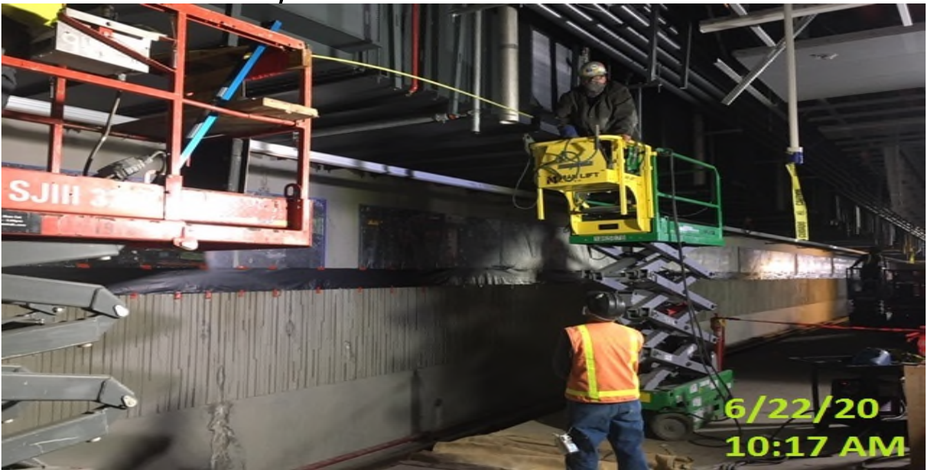
EXPO STATION – Continue welding and plumbing southbound edge light support poles along the platform level.
