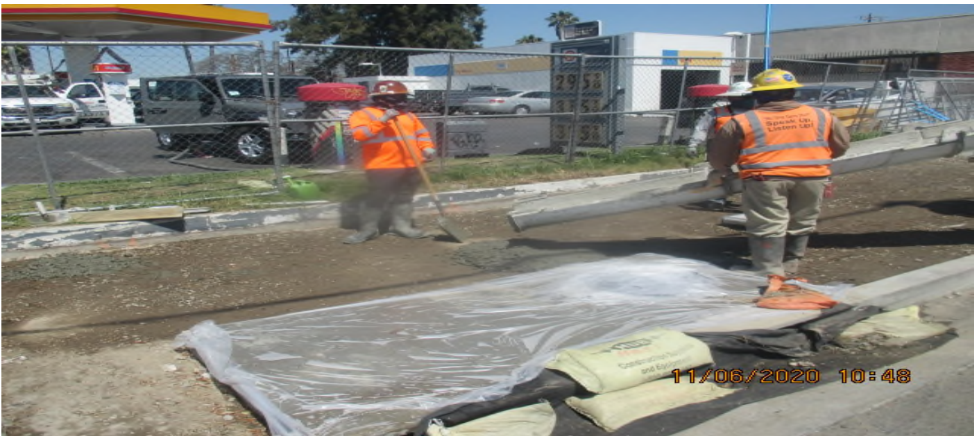
EXPO STATION – Placed concrete for sidewalk on the northwest corner of Obama Blvd and Crenshaw Blvd. 6/11/20
