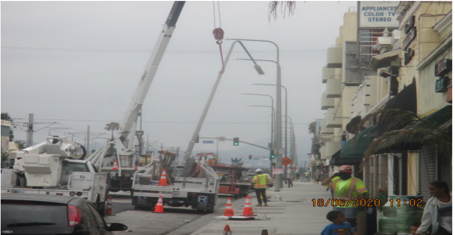
PARK MESA – Installing new permanent street light poles along northbound Crenshaw Blvd between 57th St. and 54th St. 6/18/20
