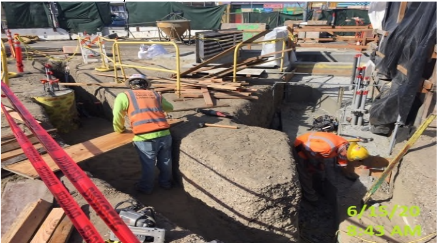
LEIMERT PARK STATION – Stripping formwork from concrete encasement of the underground trenches at the southeast section of the plaza level.
