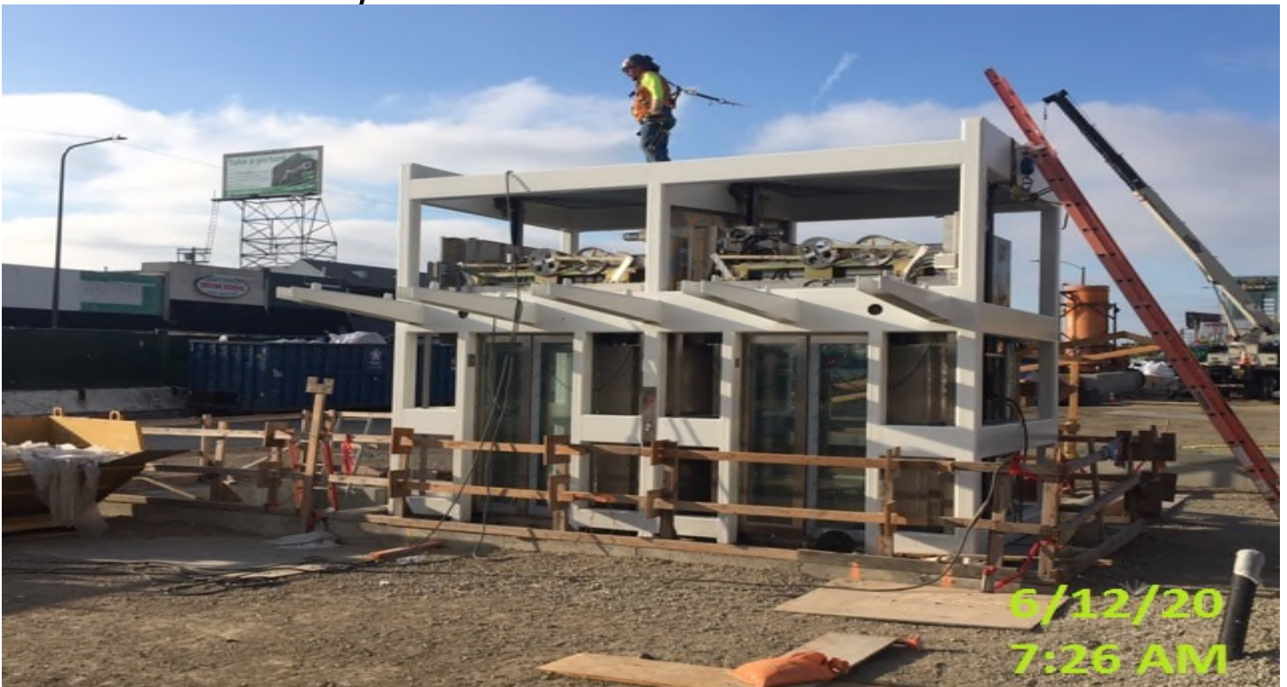
MLK STATION- WSCC Ironworkers installing metal roof deck at elevator structure #1 and #2.
