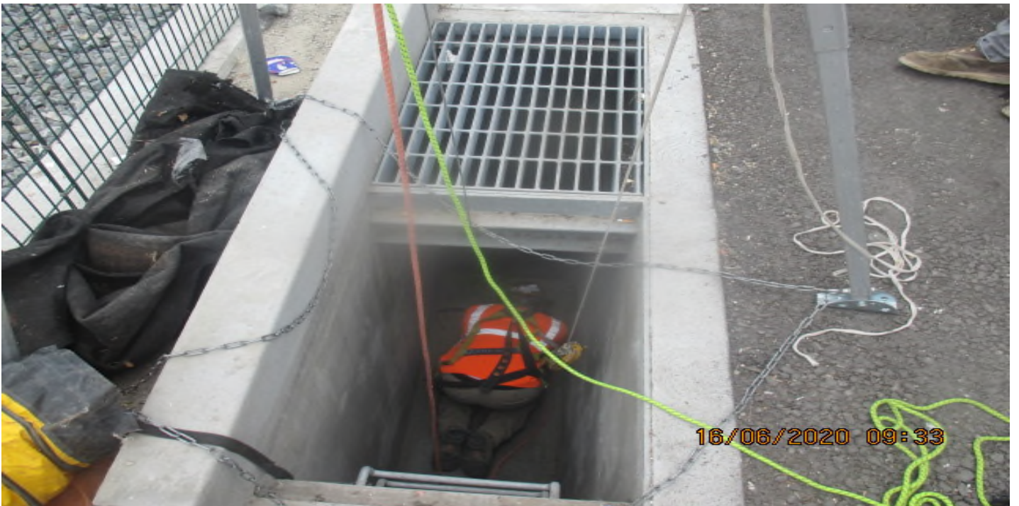
PARK MESA – Sack and patching Catch Basin #13 on southbound Crenshaw Blvd and Slauson Ave. 6/16/20
