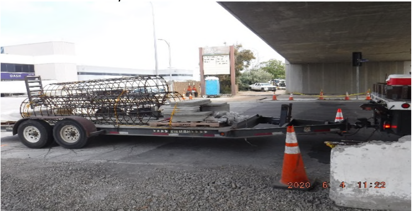
111th Street- STA 27+00 under 111th bridge looking north – DBE mobilization material & equipment.
