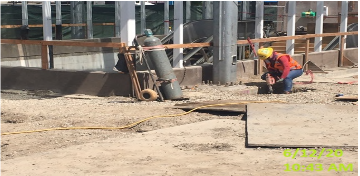
EXPO STATION – Continue excavating/trenching for underground conduit installation for landscape lighting/utilities and irrigation at the plaza level.
