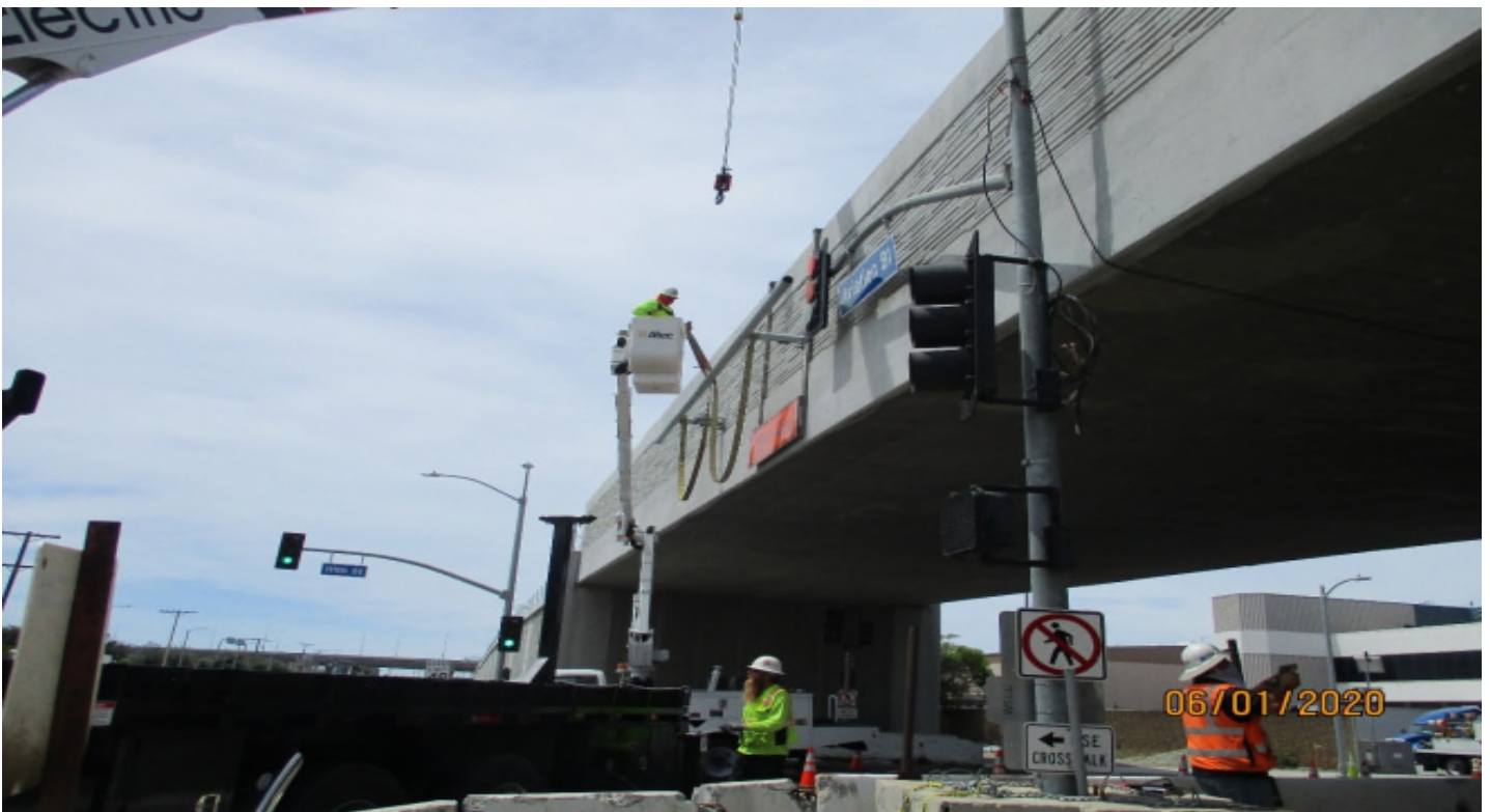
111th Street- Hanging the traffic signal mast arm at 111th street. Facing SW
