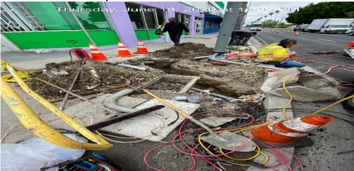
EXPO STATION – Installing conduit to supply power for the street light pole on the southwest corner of Obama Blvd and Crenshaw Blvd.
