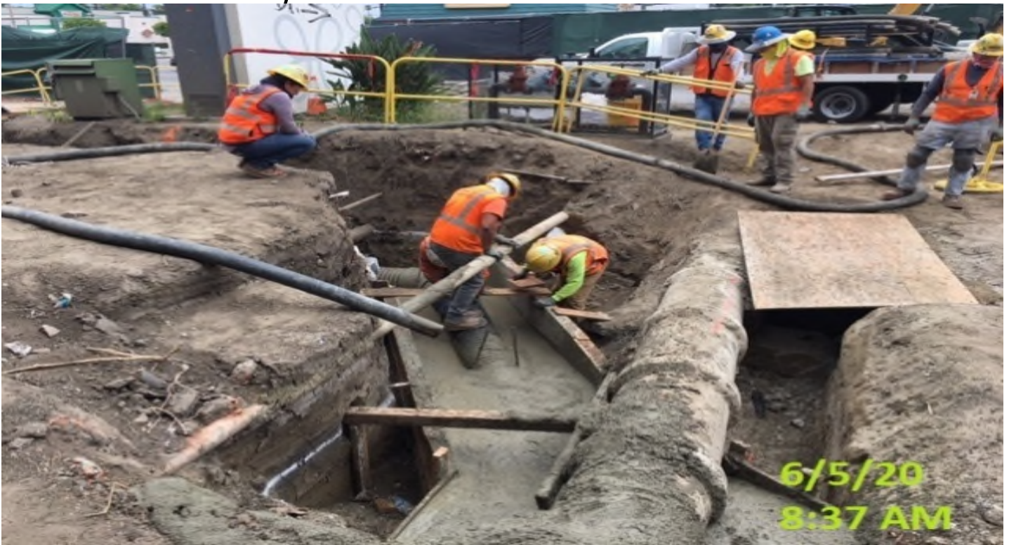
MLK – Placing slurry encasement for the 12” HDPE drainage pipe at the plaza level.
