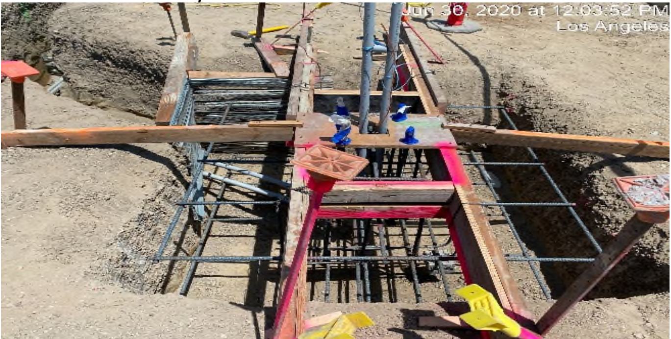
LEIMERT PARK STATION – Installing rebar for the grand pylon foundation at the southeast corner of the plaza level.
