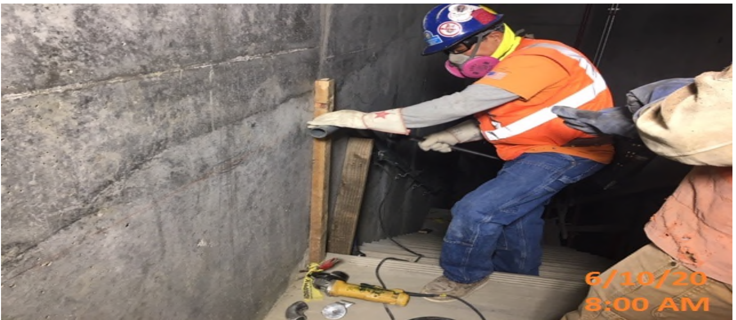
MLK STATION – Continue installing handrails at the emergency exit stairs south #2 from concourse to invert level.
