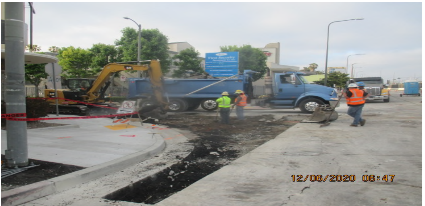
LEIMERT PARK STATION – Excavating intersection in preparation for new concrete pavement on 46th St and Leimert Blvd. 6/12/20
