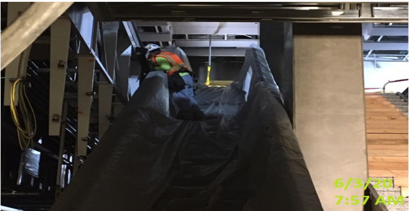
MLK STATION- VNSM crew installing stainless steel panels between escalator #4 and down stands.
