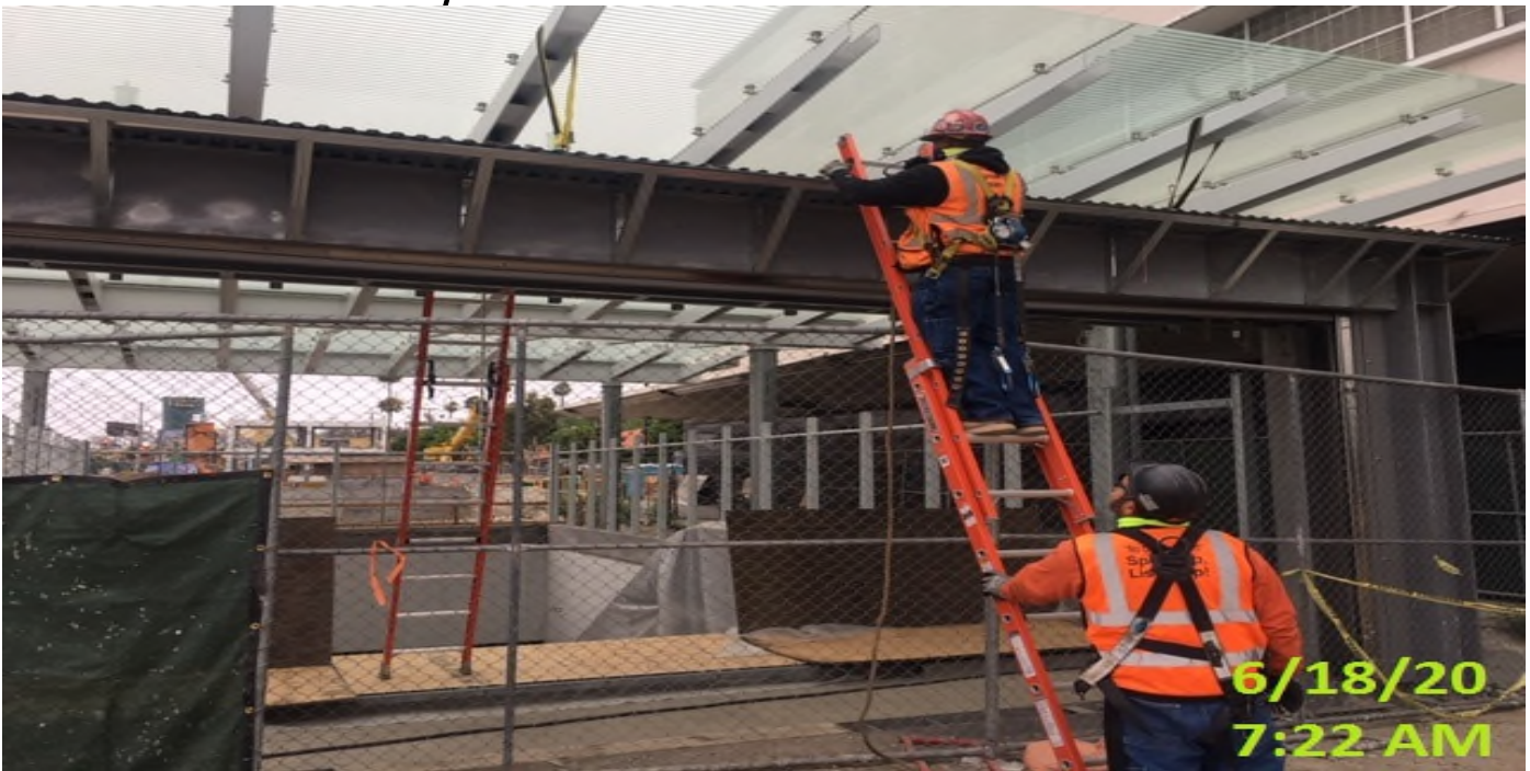
MLK STATION – Continue installing roofing deck to the main entrance canopy structure at the plaza level.
