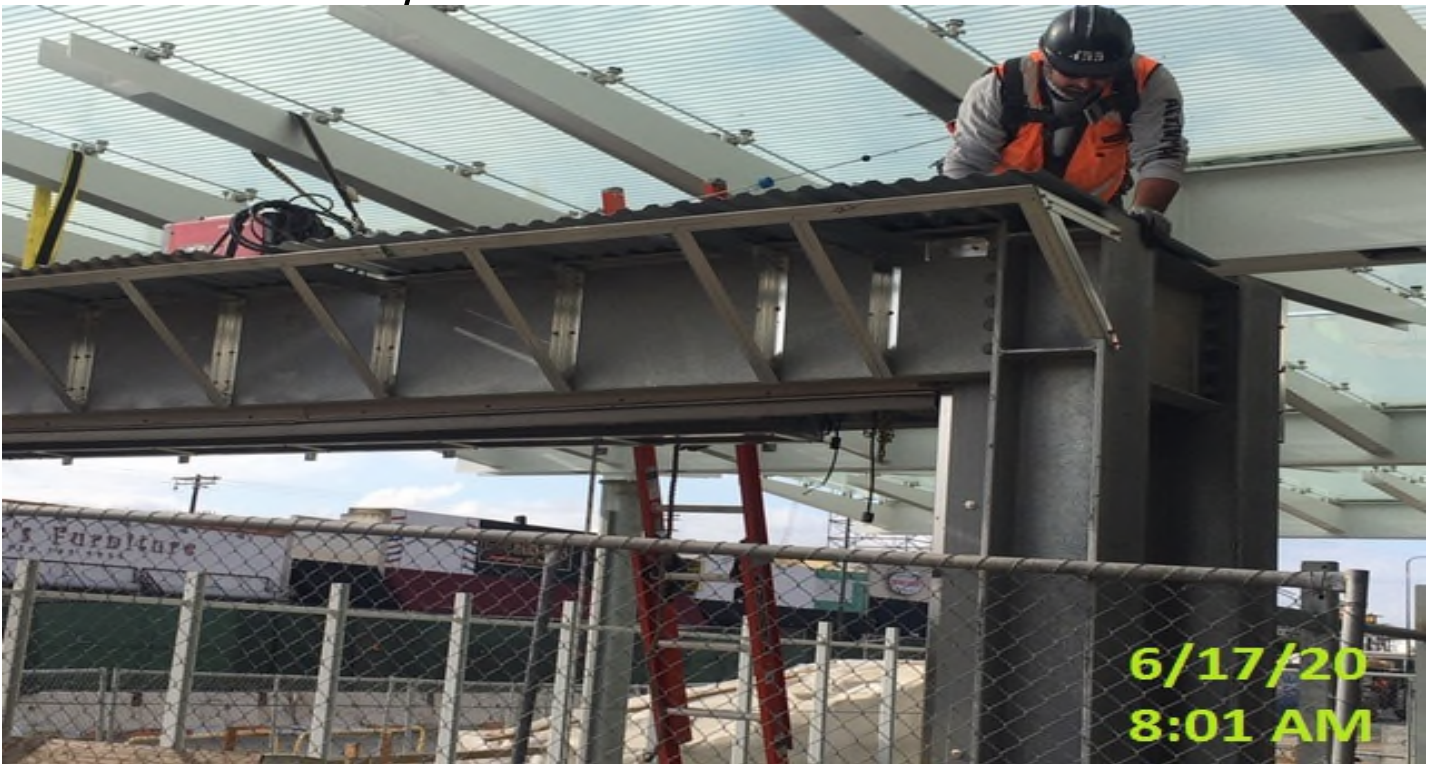
MLK - Installing roofing deck to the main entrance canopy structure at the plaza level.
