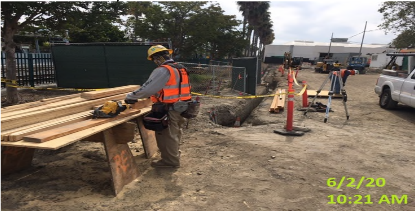
EXPO STATION – Began formwork for manhole #1 on the northwest corner of the plaza.
