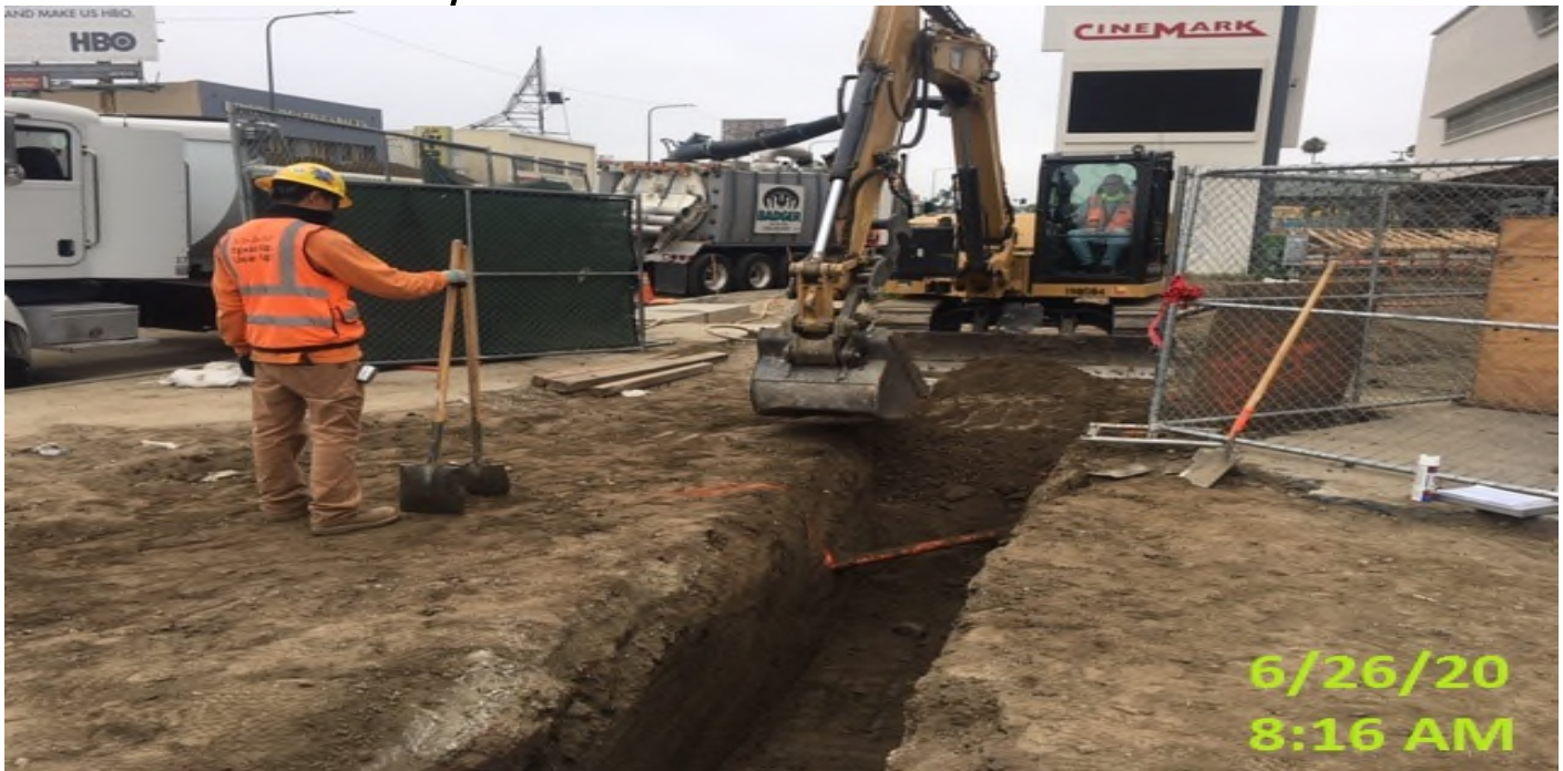
MLK STATION – Continue excavating/trenching for underground landscaping conduit installation at the west side of the plaza level.
