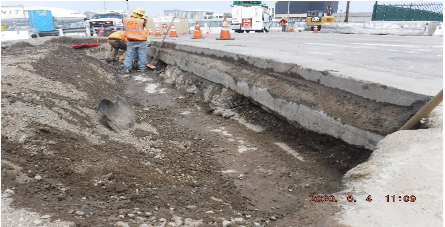
AVIATION/CENTURY- STA 55+00 at Aviation Blvd/104th St looking west – T&M work to expose DWP duct bank.
