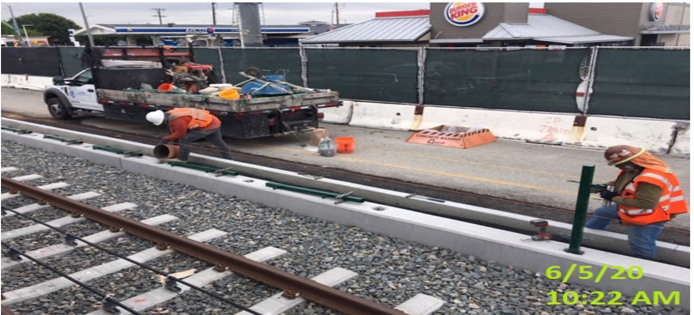
Hyde Park Station – Installing safety cables on top of the north end canopy at the platform level.
