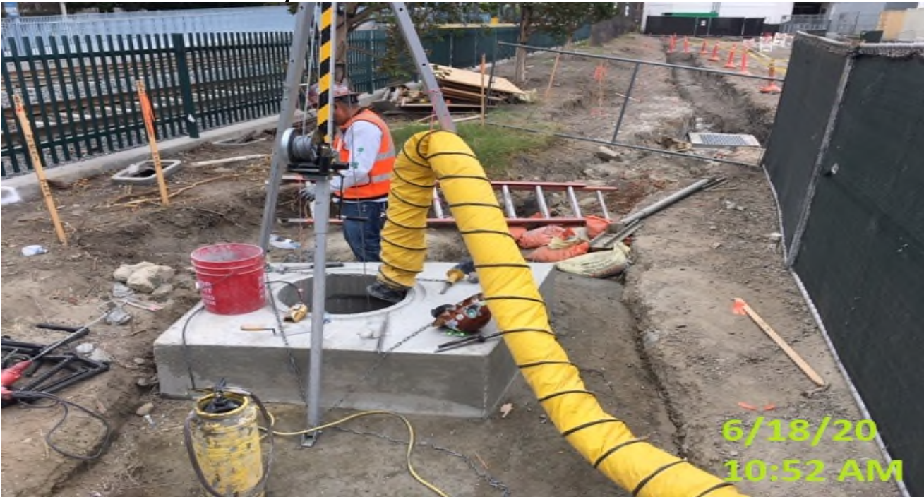
EXPO STATION – Sack and patched and installed steel steps for manhole #1 on the northwest corner of the plaza.
