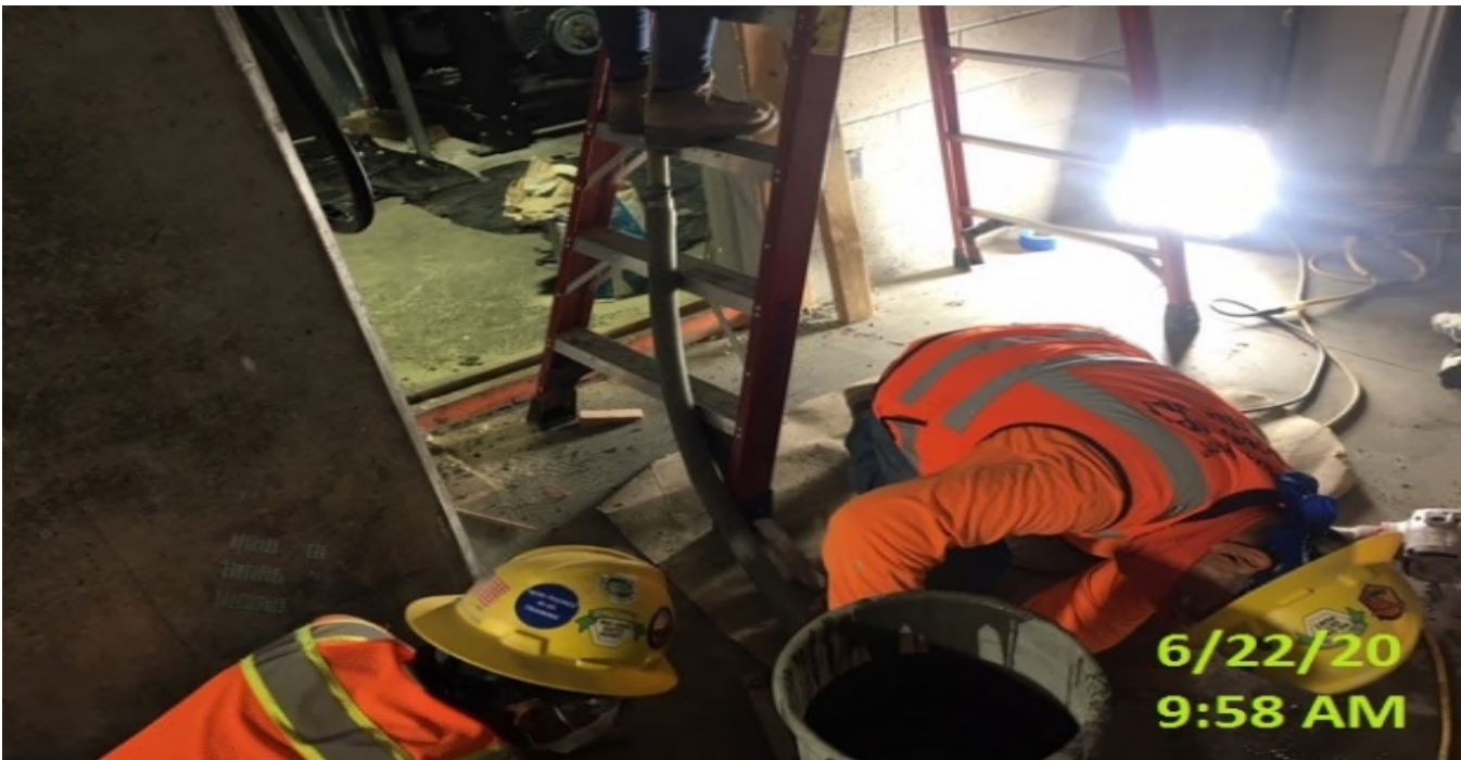
EXPO STATION – Grouting door frame for Elevator Machine Room South at the concourse level.
