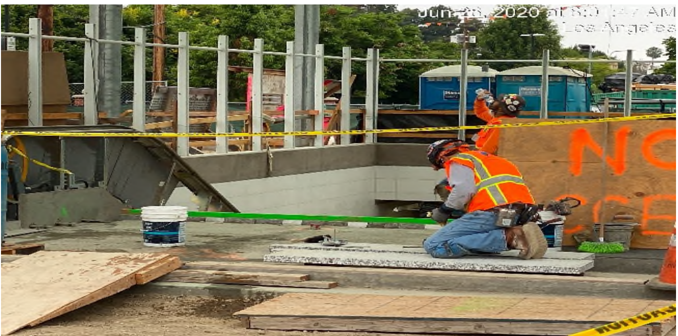
LEIMERT PARK STATION – Installing granite treads for the main entrance staircases at the plaza level.
