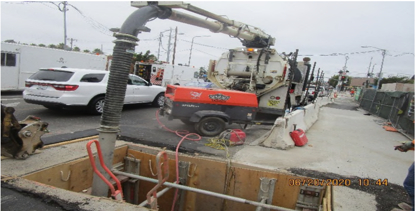
EXPO STATION- Crenshaw & (S) of Exposition Blvd, potholing for 6" ductile iron sewer vent (Pan) piping penetrations for Expo leaks.
