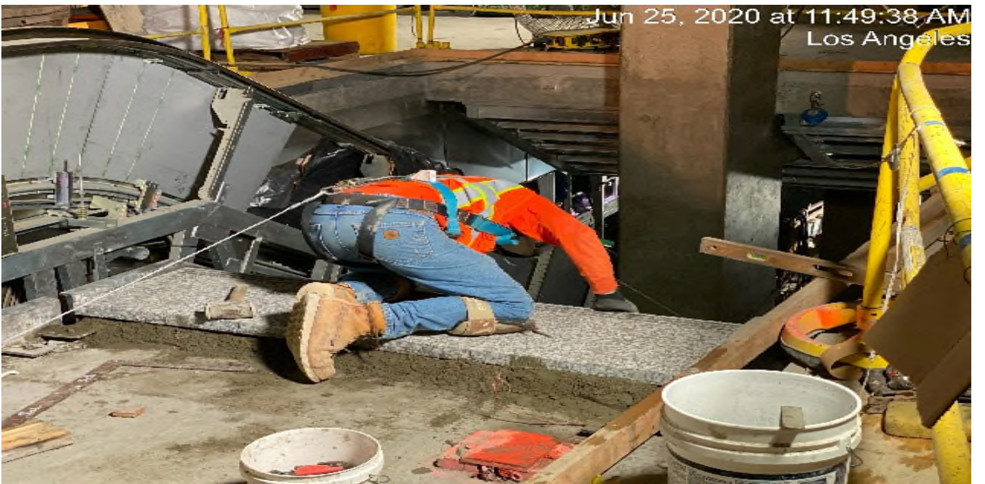
LEIMERT PARK STATION – Continue installing granite riser and threads for staircase #3 from concourse to platform level.
