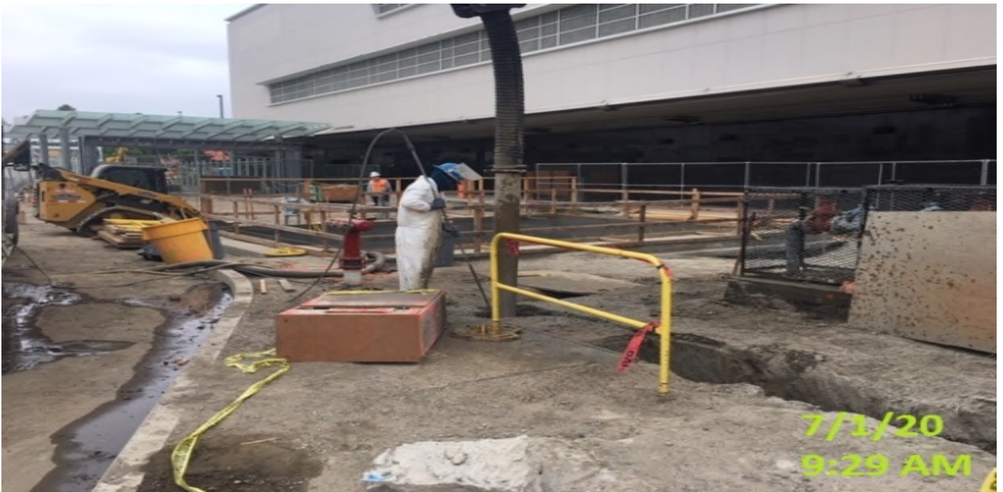
MLK STATION – Resume trenching/potholing for underground landscaping conduit installation at the northwest corner of the plaza level.
