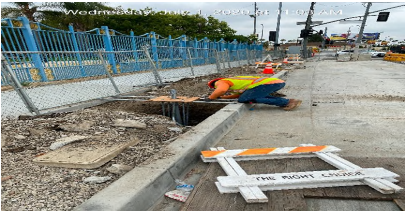
LEIMERT PARK STATION – Installing pedestrian signal head foundations on northbound Crenshaw Blvd between Vernon Ave and 43rd Pl.
