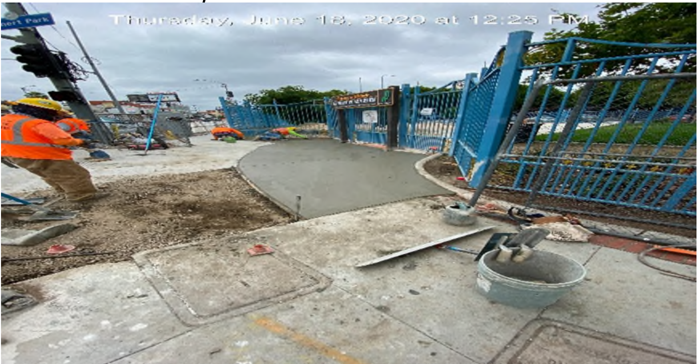
LEIMERT PARK STATION – Placed concrete for sidewalk on the northeast corner of Vernon Ave and Crenshaw Blvd.
