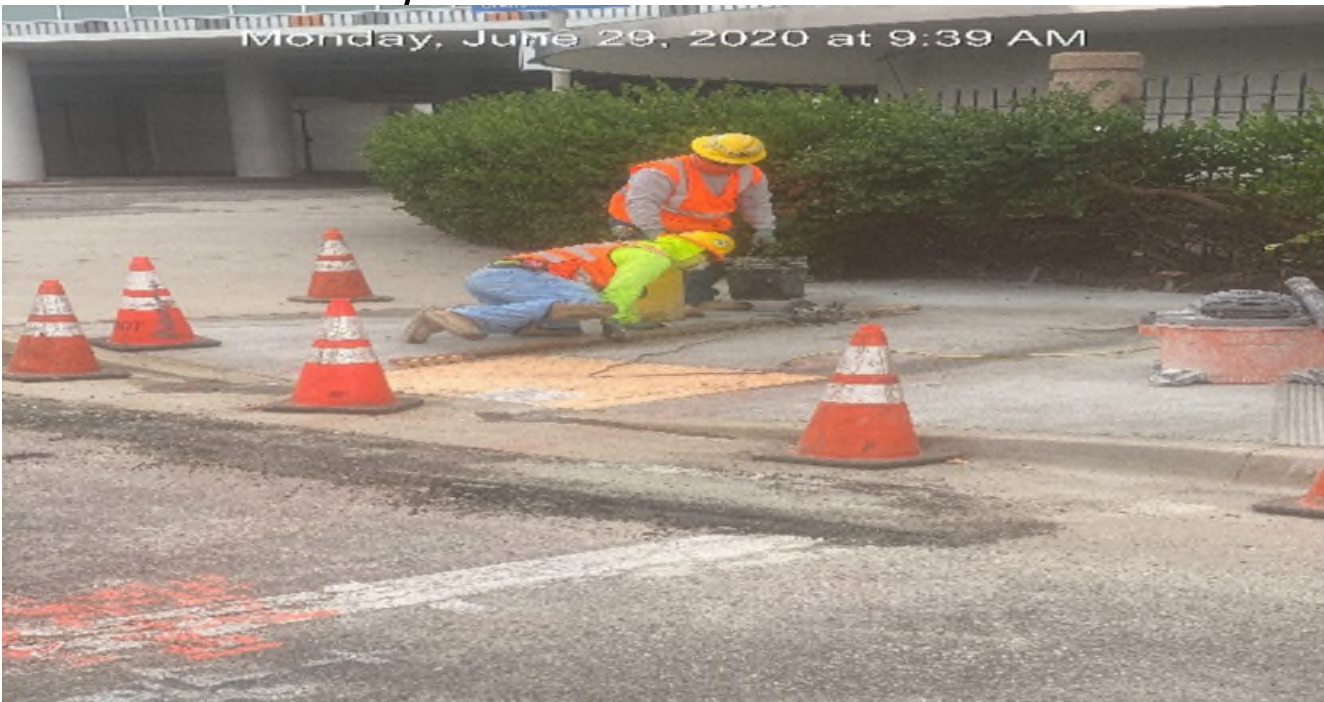
MLK STATION – Saw cutting new ADA ramp and curb/gutter on the northwest corner of MLK Blvd and Crenshaw Blvd.
