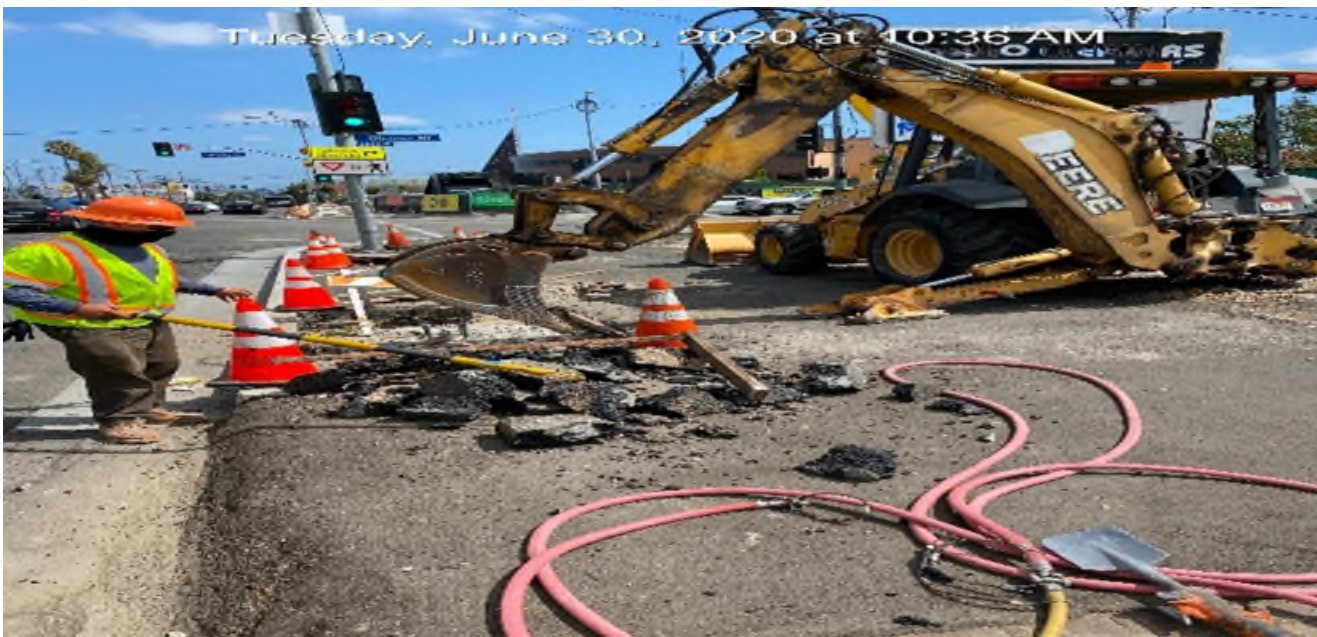
EXPO STATION – Excavating for new pedestrian signal head foundations on Crenshaw Blvd between Rodeo Rd and Obama Blvd.
