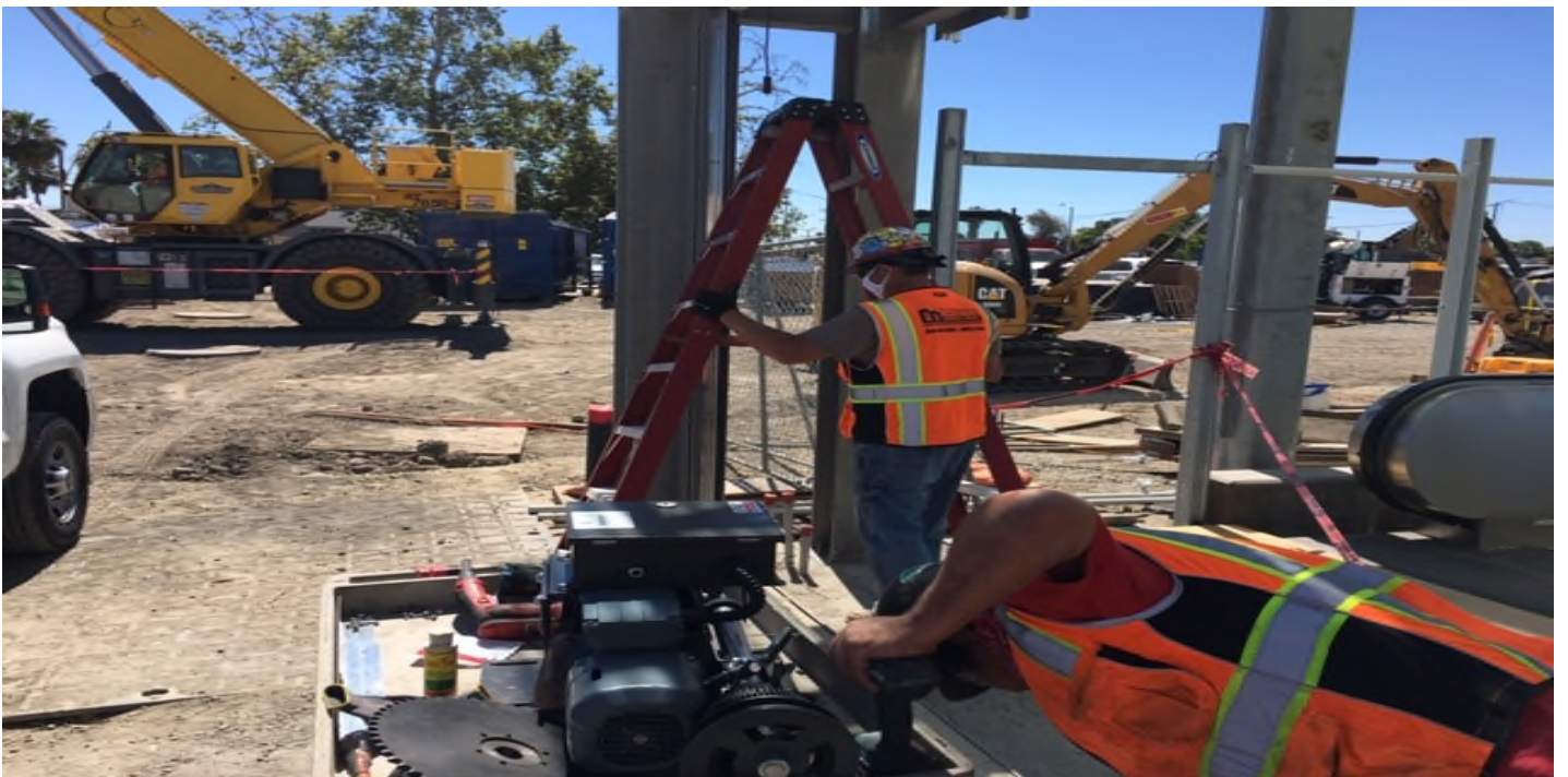
EXPO STATION – Installing motor for the overhead coiling grille for the main entrance canopy at the plaza level.
