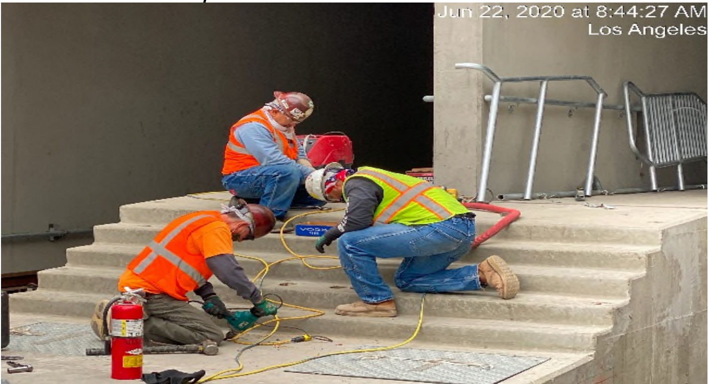
UG4 – Installing handrails at the south end portal and throughout the northbound tunnel.
