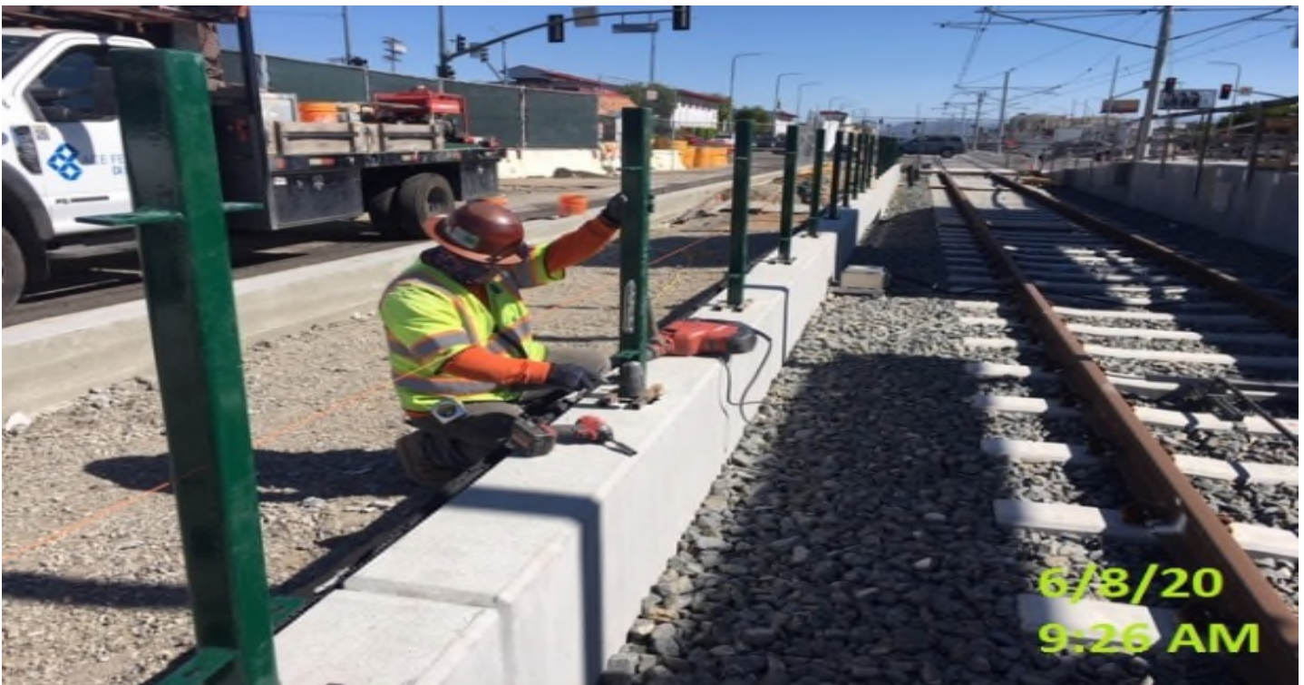
Hyde Park Station – Continue installing guardrail posts along the guideway curb on the southbound track.
