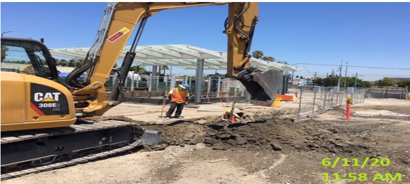
EXPO STATION – Continue excavating/trenching for underground conduit installation for landscape lighting/utilities and irrigation at the plaza level.
