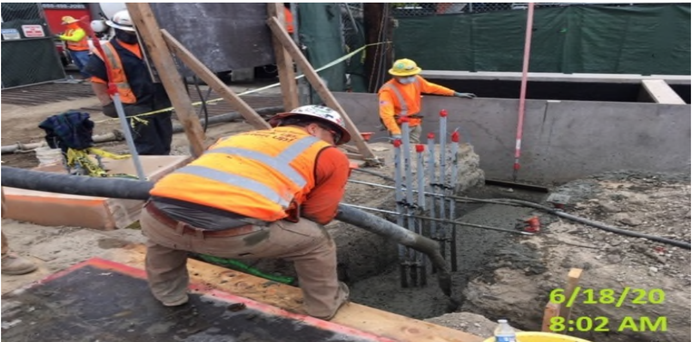
LEIMERT PARK STATION – Placing concrete inside trenches for underground conduit at the plaza level.
