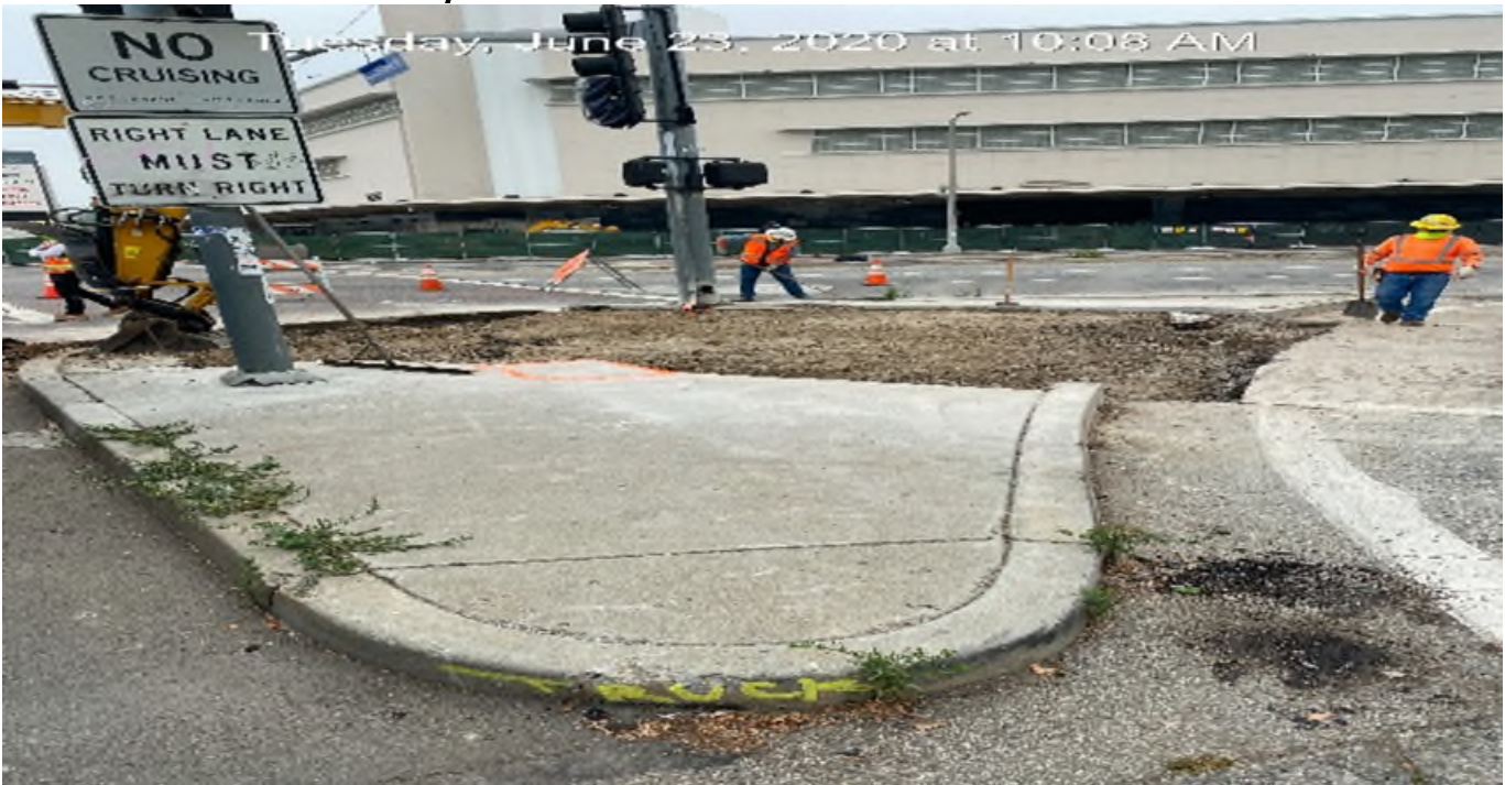
MLK STATION – Excavating/demolishing for new ADA ramp and sidewalk installation on the west median corner of MLK Blvd and Crenshaw Blvd.
