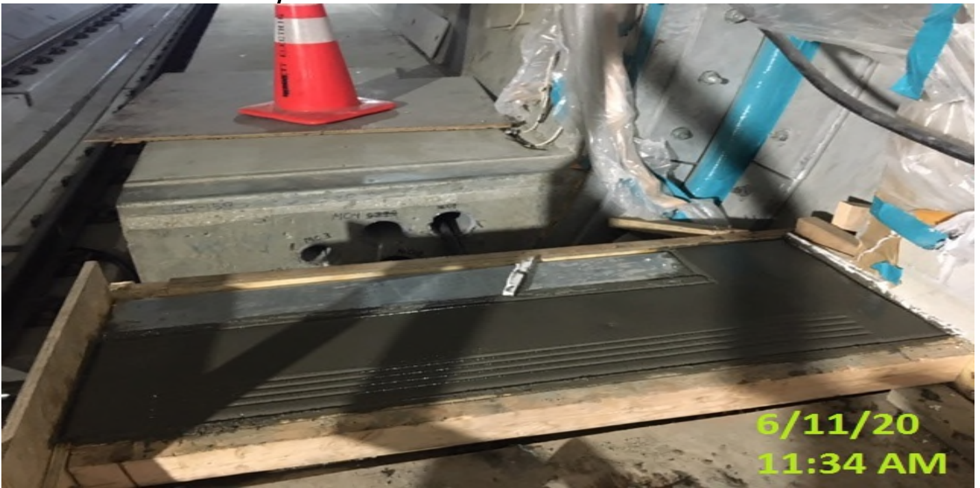
EXPO STATION- WSCC crew encasing embed in concrete for stair landing at emergency walkway.
