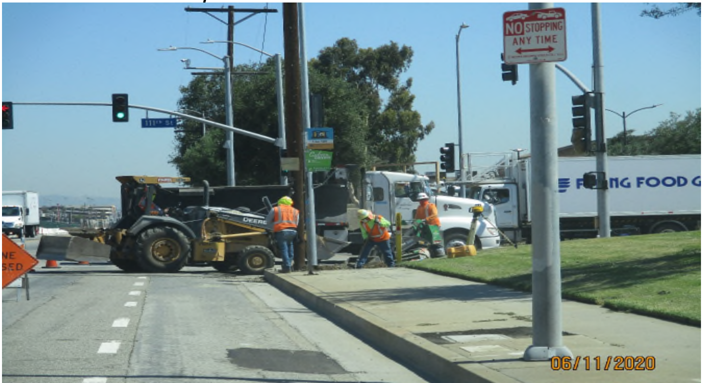
111th Street- Grading and base placement for the ADA ramps at 111th street. Facing north.
