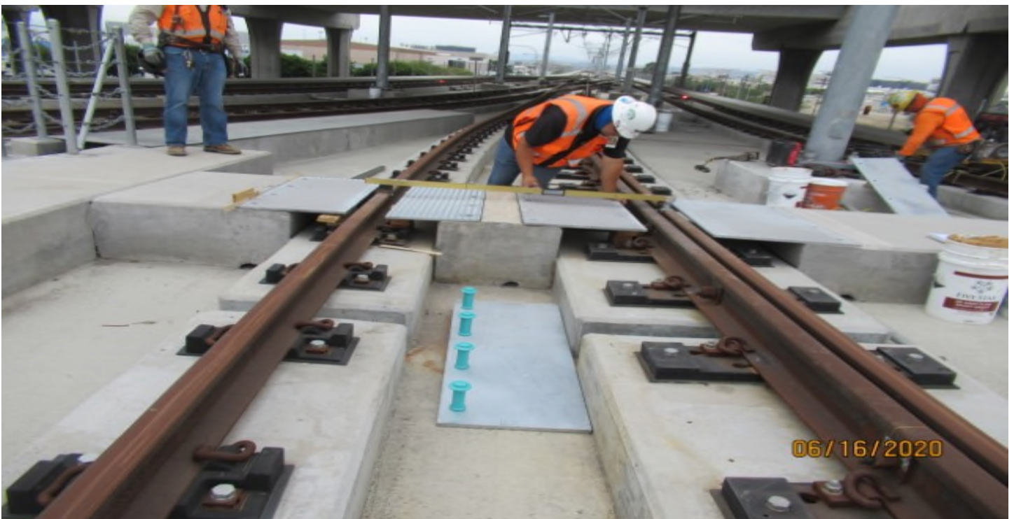
GREENLINE UNDERPASS- WSCC QC inspector checking cross level & track gauge where crossing plates will be re-installed GL Wye (looking north) Rework.
