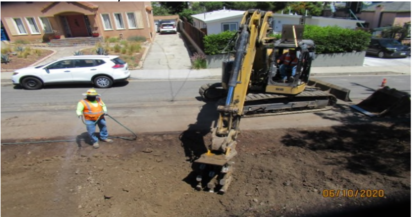
La Brea – WSCC dirt crew rolling slope & adjusting elevations at La Brea (looking west)
