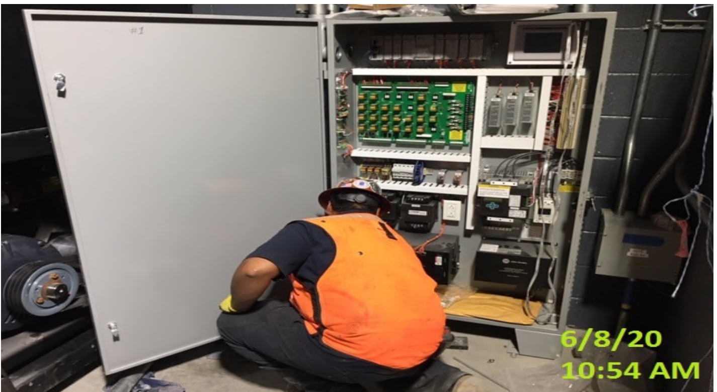
EXPO STATION- Excelsior running lines from motor leads to control panel.
