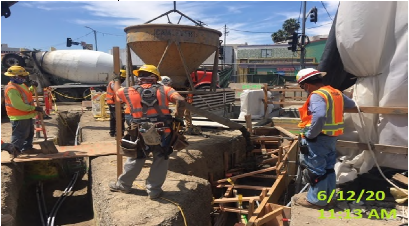
LEIMERT PARK STATION – Placing concrete for underground conduit trenches at the southeast section of the plaza level.
