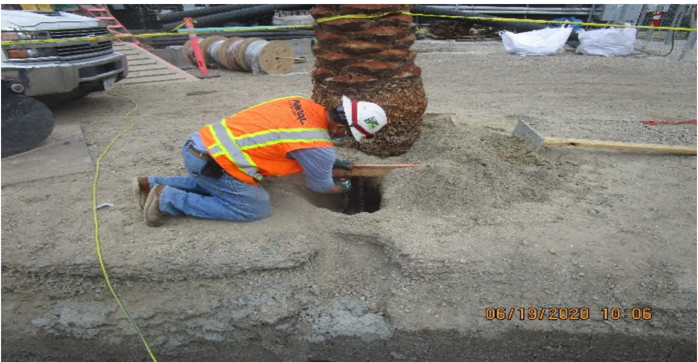
LEIMERT PARK STATION – Continue underground conduit installation for landscape lighting and utilities at the plaza level.
