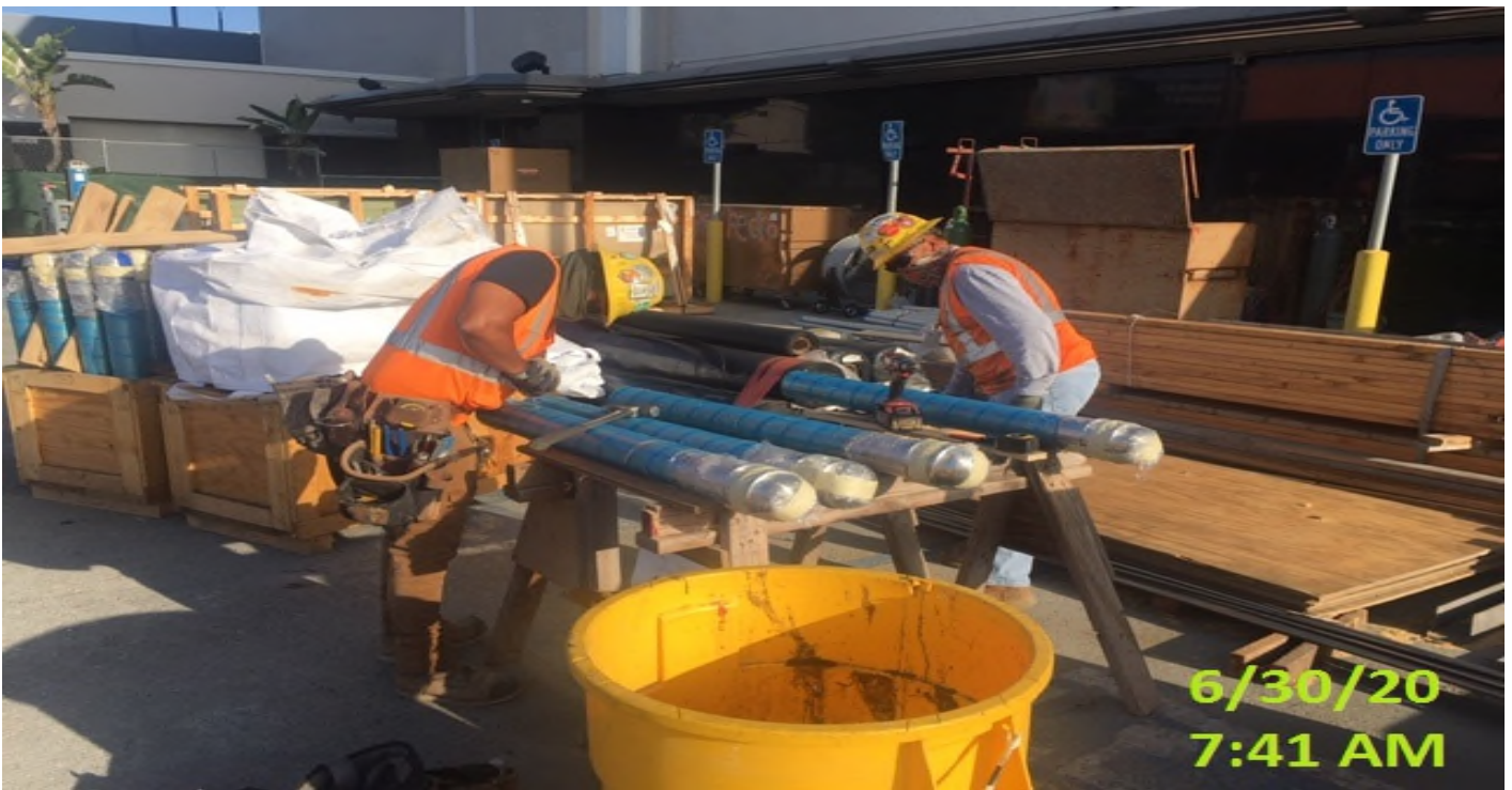
MLK STATION – Drilling and tapping the stainless steel bollards for ground wire prior to installation at the plaza level.
