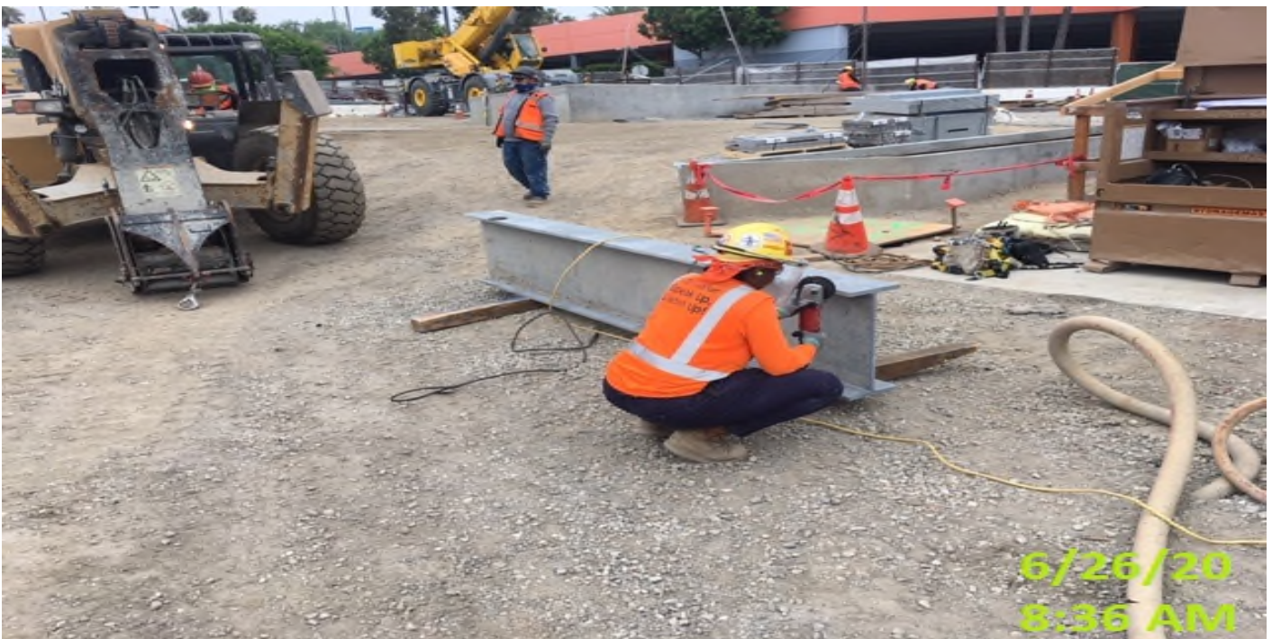
MLK STATION – Installing beams to the south air exhaust vent shaft and continue steel grating installation at the plaza level.
