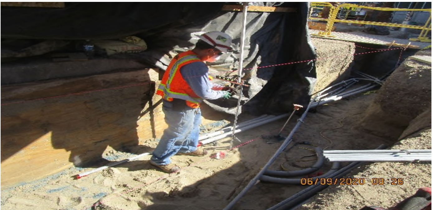
LEIMERT PARK STATION – Continue underground conduit installation for landscape lighting and utilities at the plaza level.
