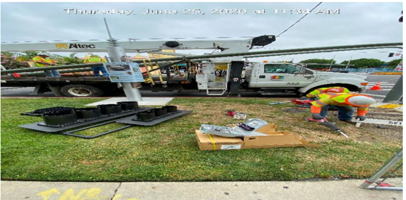
LEIMERT PARK STATION – Preparing to install street light pole on the southwest corner of Vernon Ave and Crenshaw Blvd.
