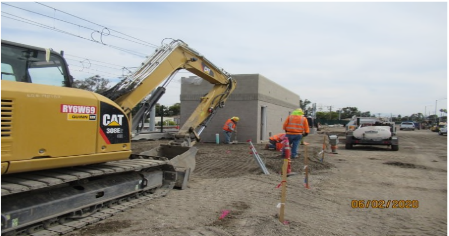
La Brea – WSCC dirt crew installing pad for future concrete at La Brea station (looking northwest)
