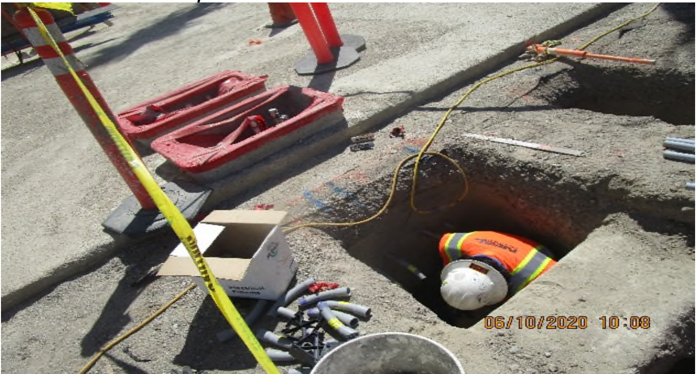
VERNON STATION- Continued rough in underground CCTV & power (JB-38-175D & JB-76-775D) to 18"x18"x8" PB's.
