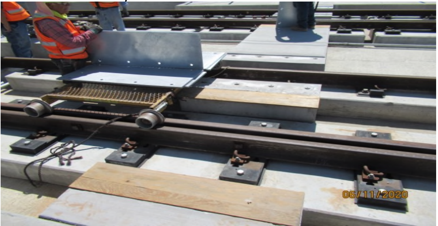
GREENLINE UNDERPASS- WSCC re-installing emergency walkway plates on west leg of GL Wye.
