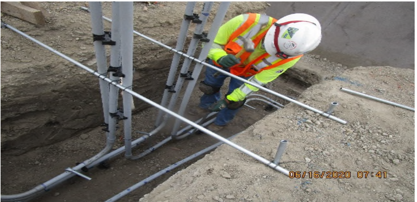
LEIMERT PARK STATION – Continue underground conduit installation for landscape lighting and utilities at the plaza level.
