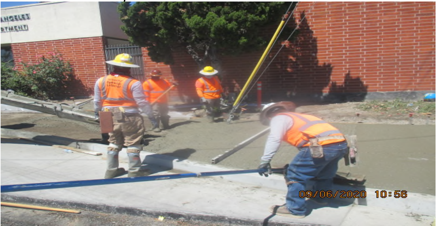
EXPO STATION – Placed concrete for sidewalk on southbound Crenshaw Blvd between Exposition Blvd and Obama Blvd. 6/9/20
