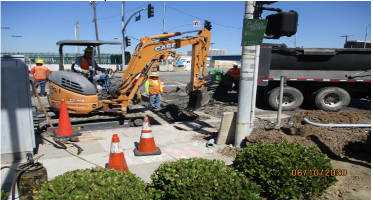
104th Street- Removal of the temporary AC for the traffic signal trench at 104th street. Facing
