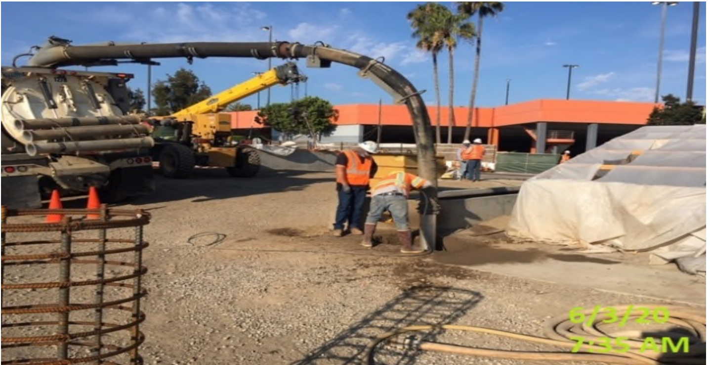
MLK Station - Potholing for the installation of light pole foundations at the plaza level.
