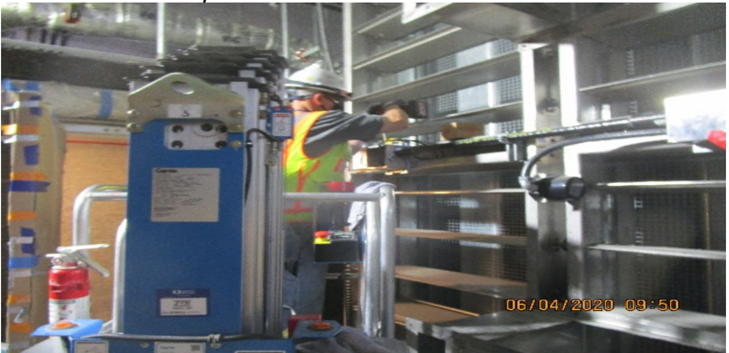
VERNON STATION- Tunnel vent plenum (N) C125 TFD-6-302 Begin installing breathers & drains at Nema4X pull boxes.
