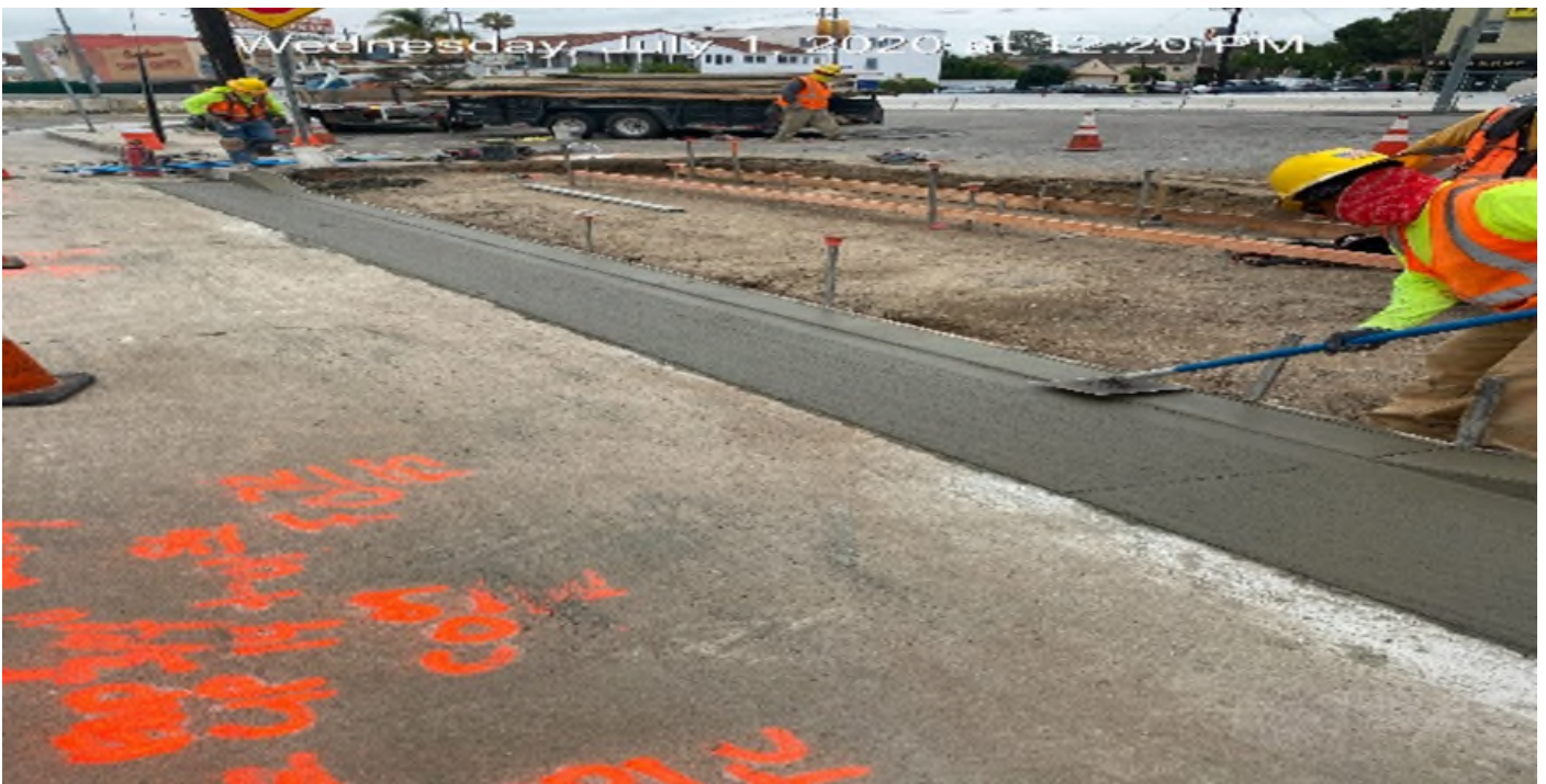
LEIMERT PARK STATION – Placing concrete for new curb/gutter and driveway installation at southbound Leimert Blvd and Crenshaw Blvd.
