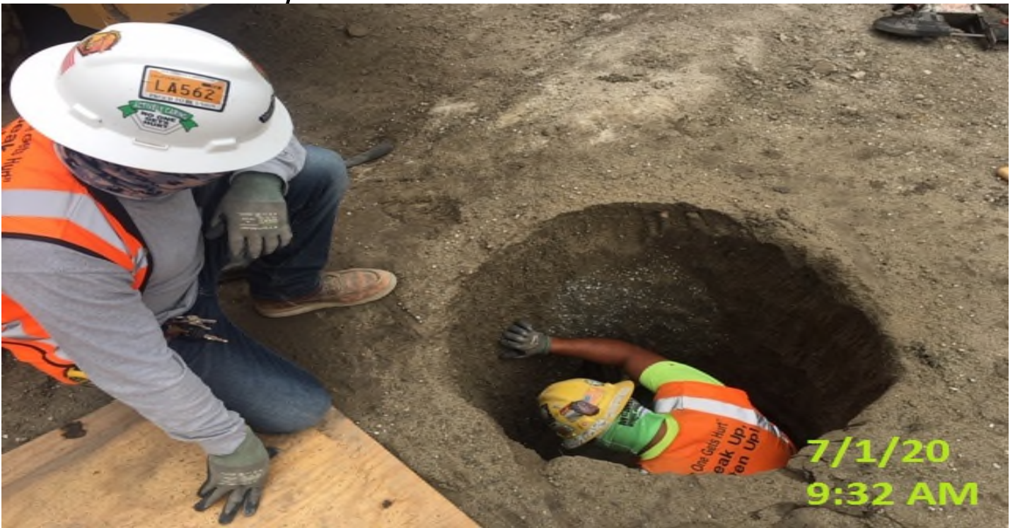
MLK STATION – Continue setting rebar cages for pedestrian light pole foundations throughout the plaza level.
