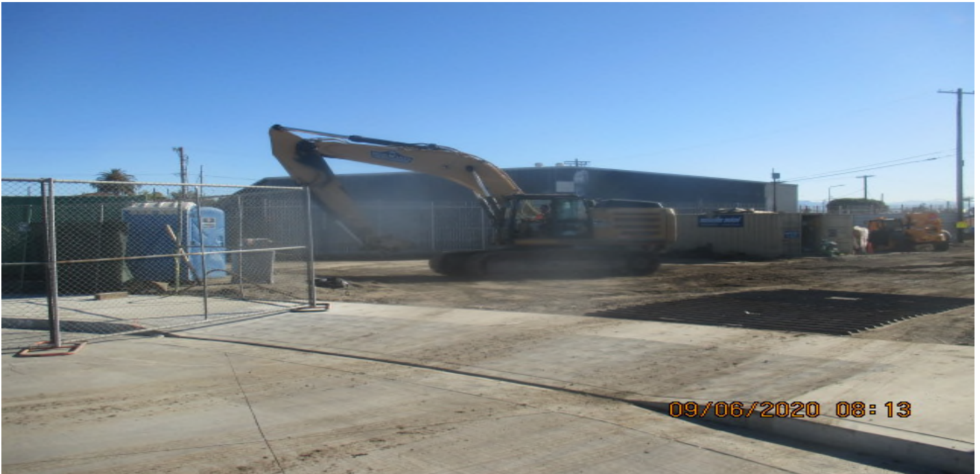
UG3 – Continue grading the north east section of Victoria Yard for upcoming pavement installation. 6/9/20
