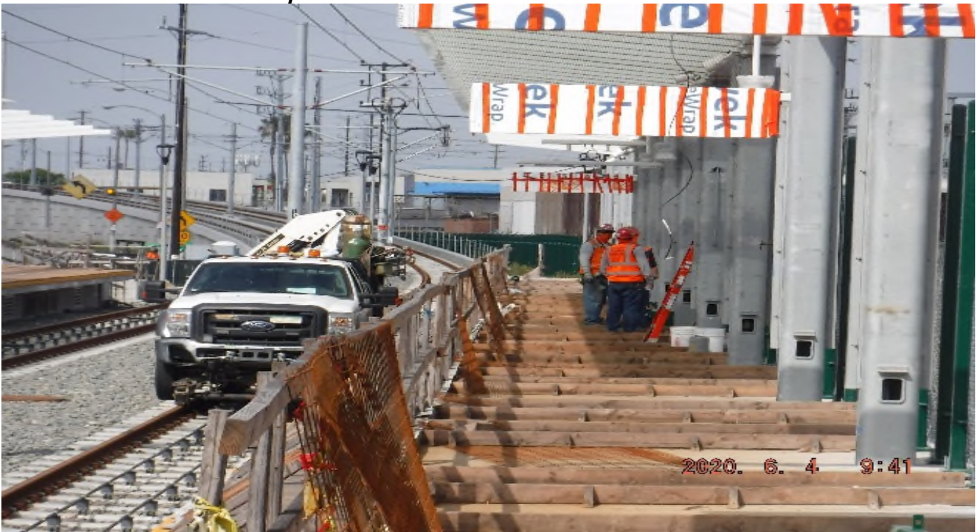
Hindry Station – STA 135+00 TK#3/SB looking south – Hindry Station install the 8' fence posts along the backside of the platform.
