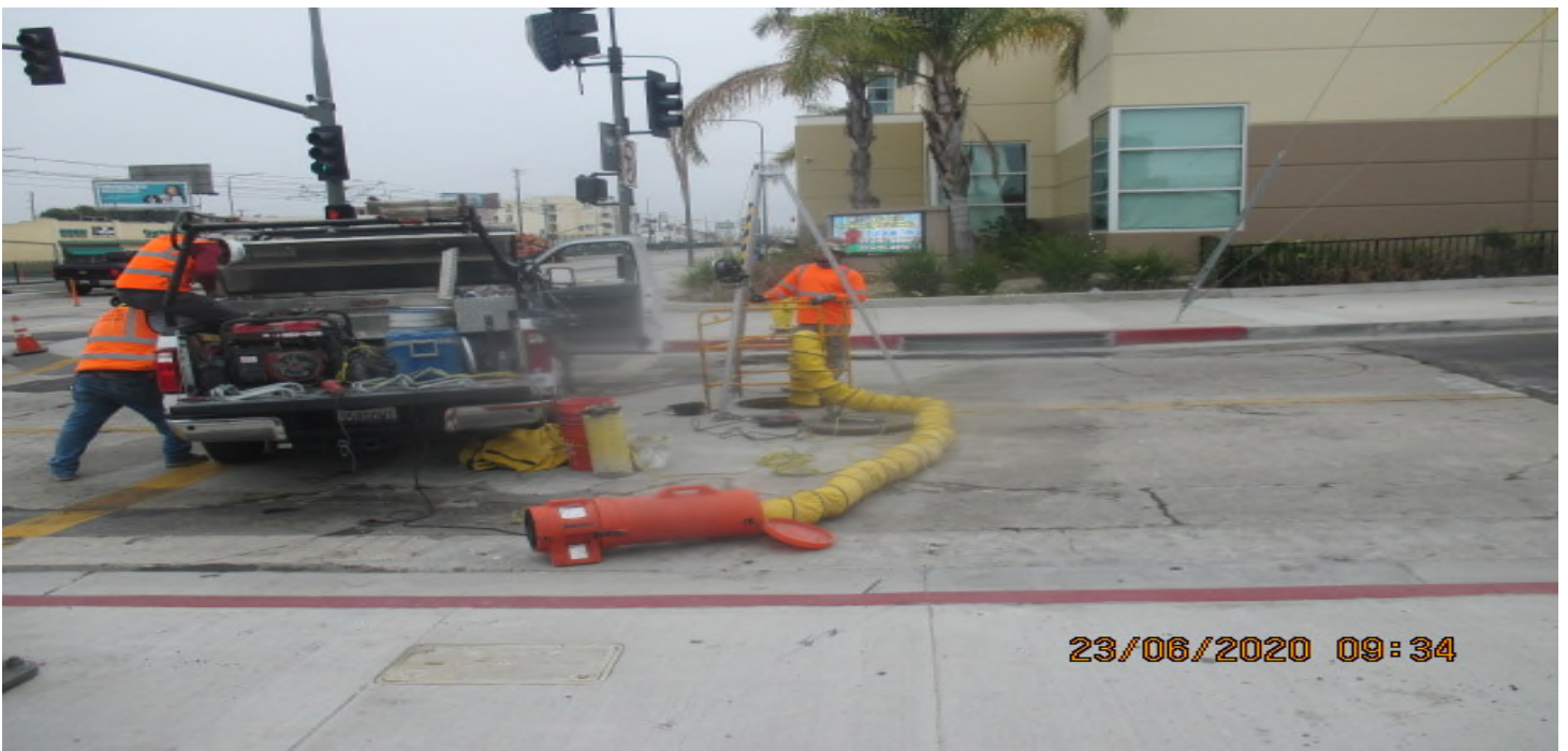
PARK MESA – Sack and patching Manhole #23 on southbound Crenshaw Blvd and 52nd St. 6/23/20
