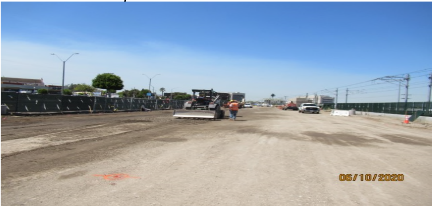
La Brea – WSCC adjusting elevations on CMB in La Brea parking lot, using front end skip loader (looking south)
