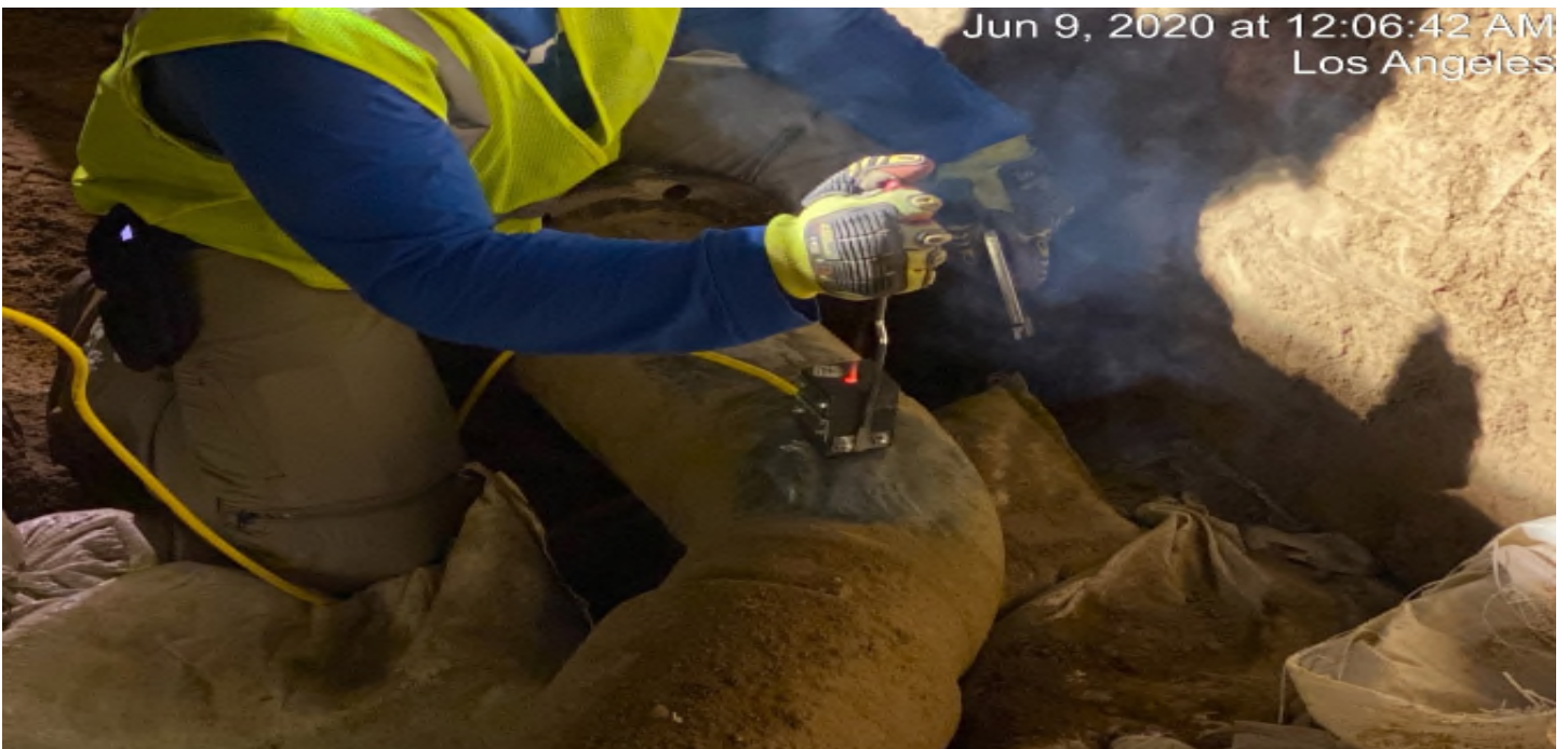
AVIATION/CENTURY- CorPro installing Cathodic Protection for 8” fire line at Aviation and 104 th
