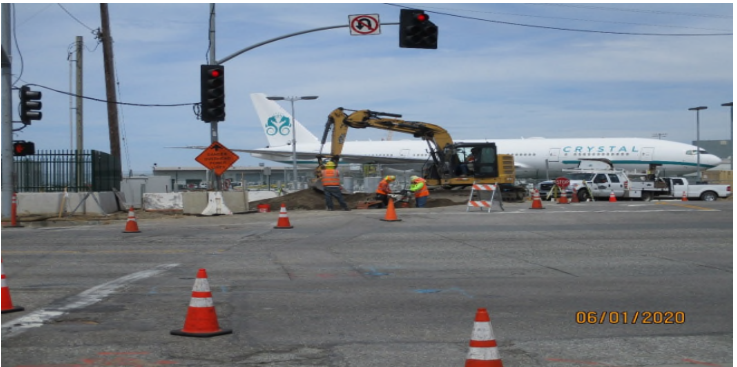
104th Street- Over-excavation and compaction of the sidewalk subgrade at 104th street. Facing west.
