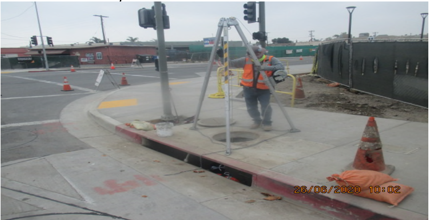
PARK MESA – Sack and patching Catch Basin #31 on the southwest corner of 67th St & Crenshaw Blvd. 6/26/20
