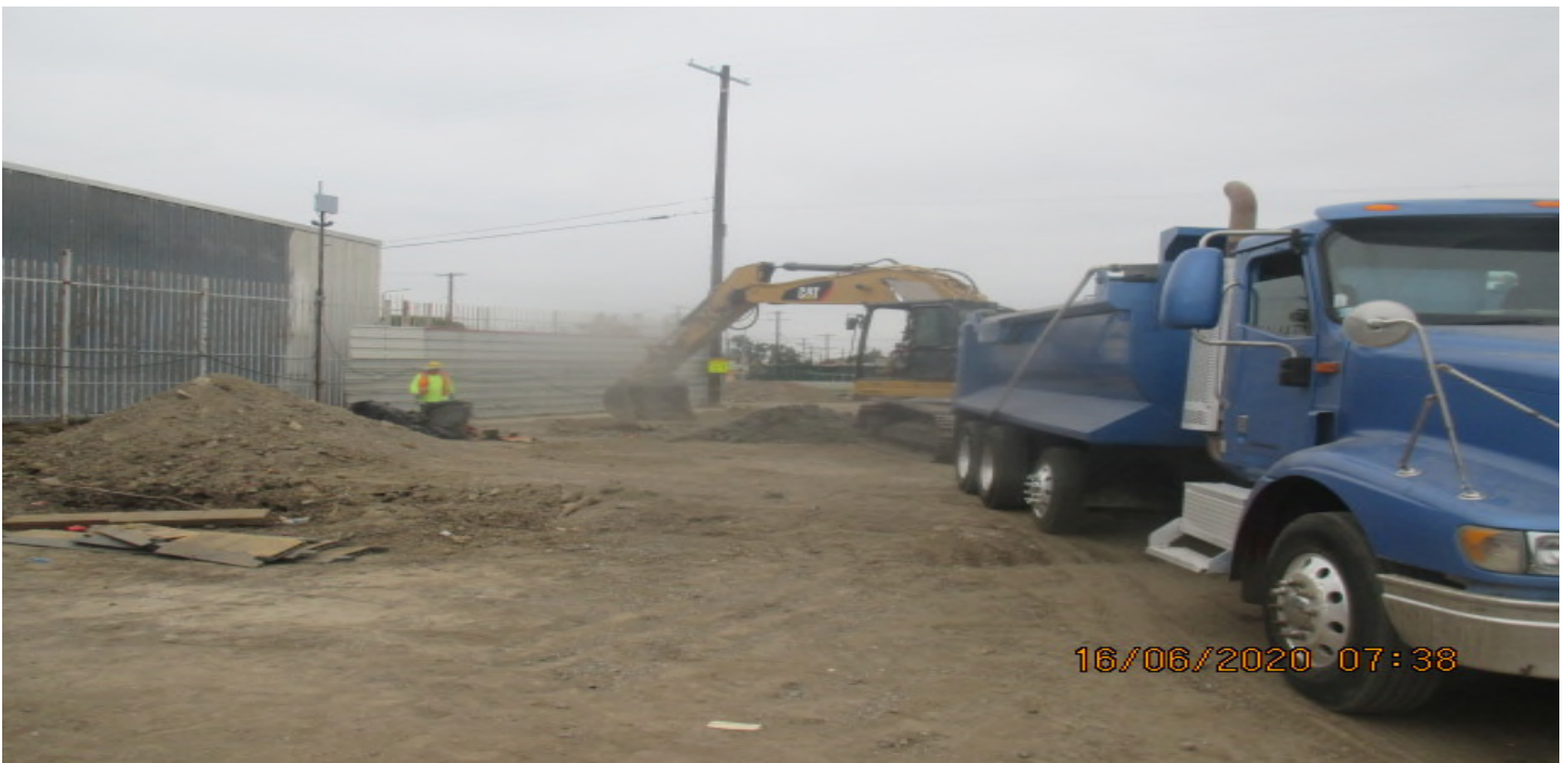
UG3 – Continue excavating/grading the north east section of Victoria Yard for upcoming pavement installation. 6/16/20
