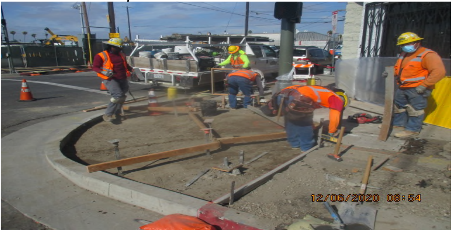
PARK MESA – Installing block-out forms for concrete placement of ADA ramp on the northwest corner of 67th St & Crenshaw Blvd. 6/12/20
