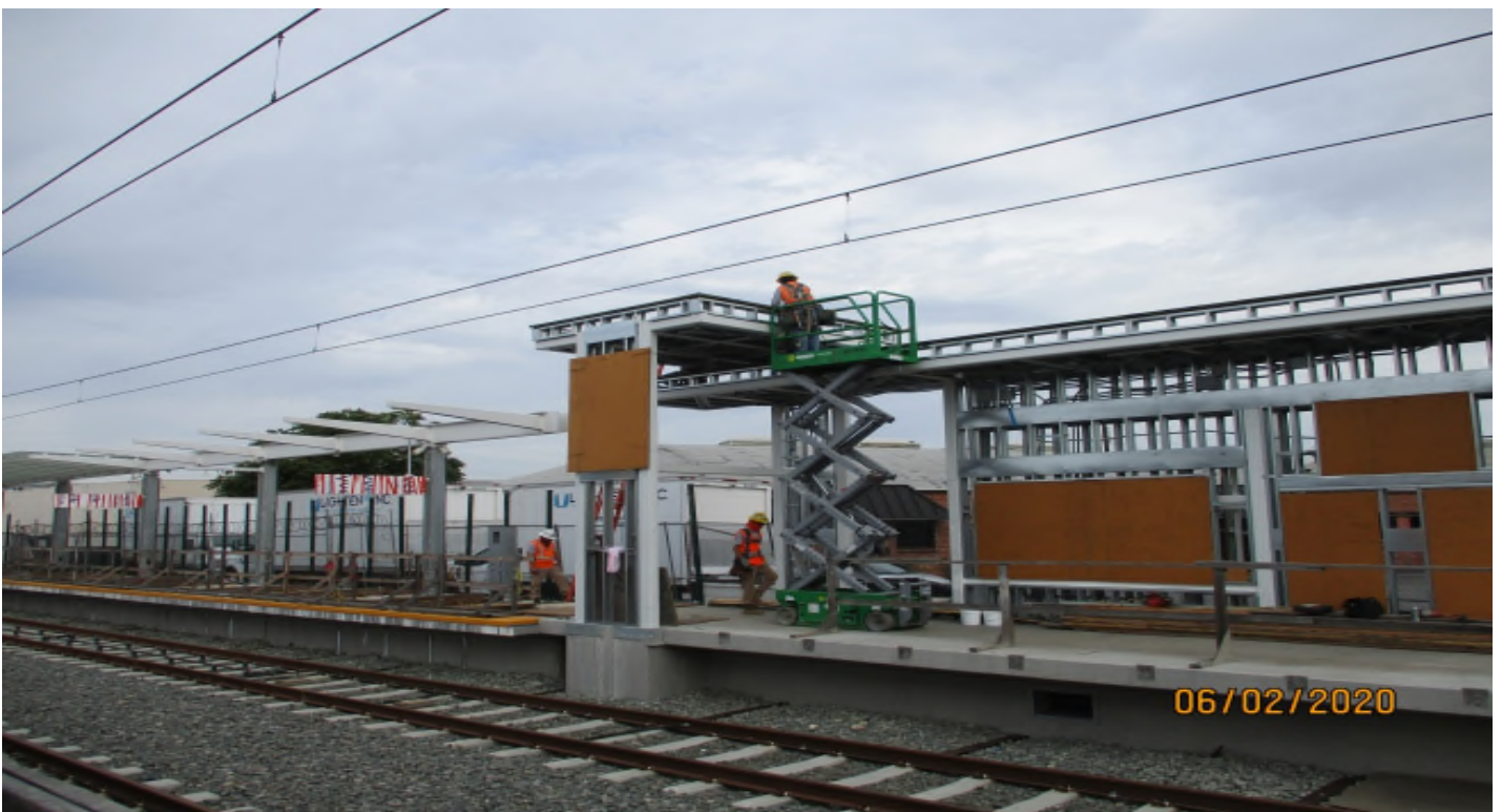
Hindry Station – Framing for the TVM roof deck at the Hindry Station SB platform.
