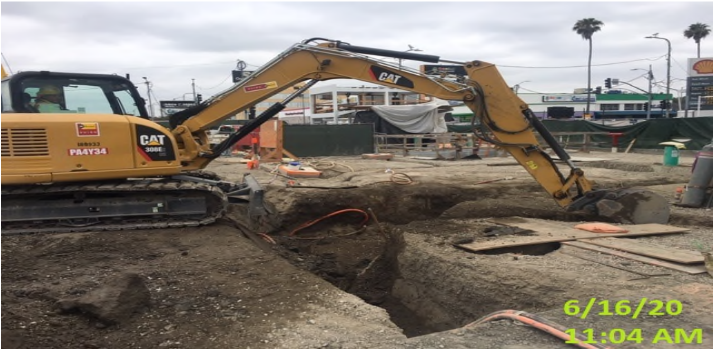
EXPO STATION – Continue excavating/trenching for underground conduit installation for landscape lighting/utilities and irrigation at the plaza level.
