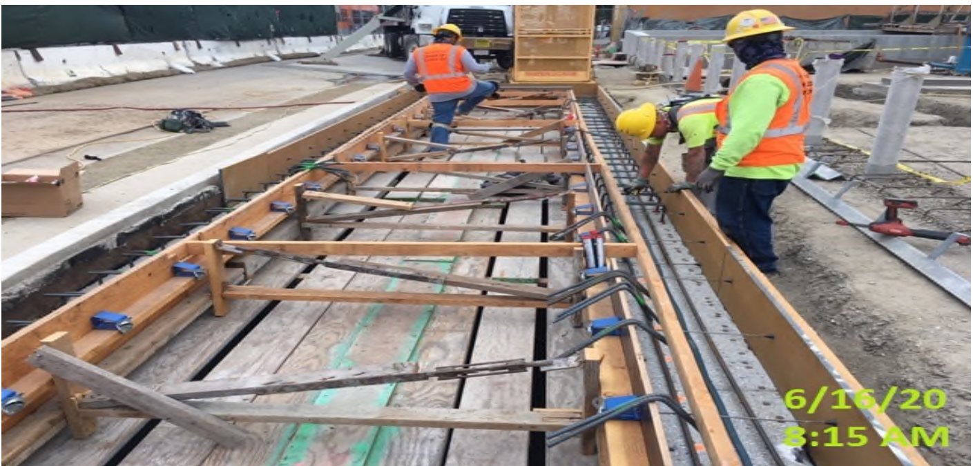
LEIMERT PARK STATION – Building formwork for the air exhaust shaft at the plaza level.
