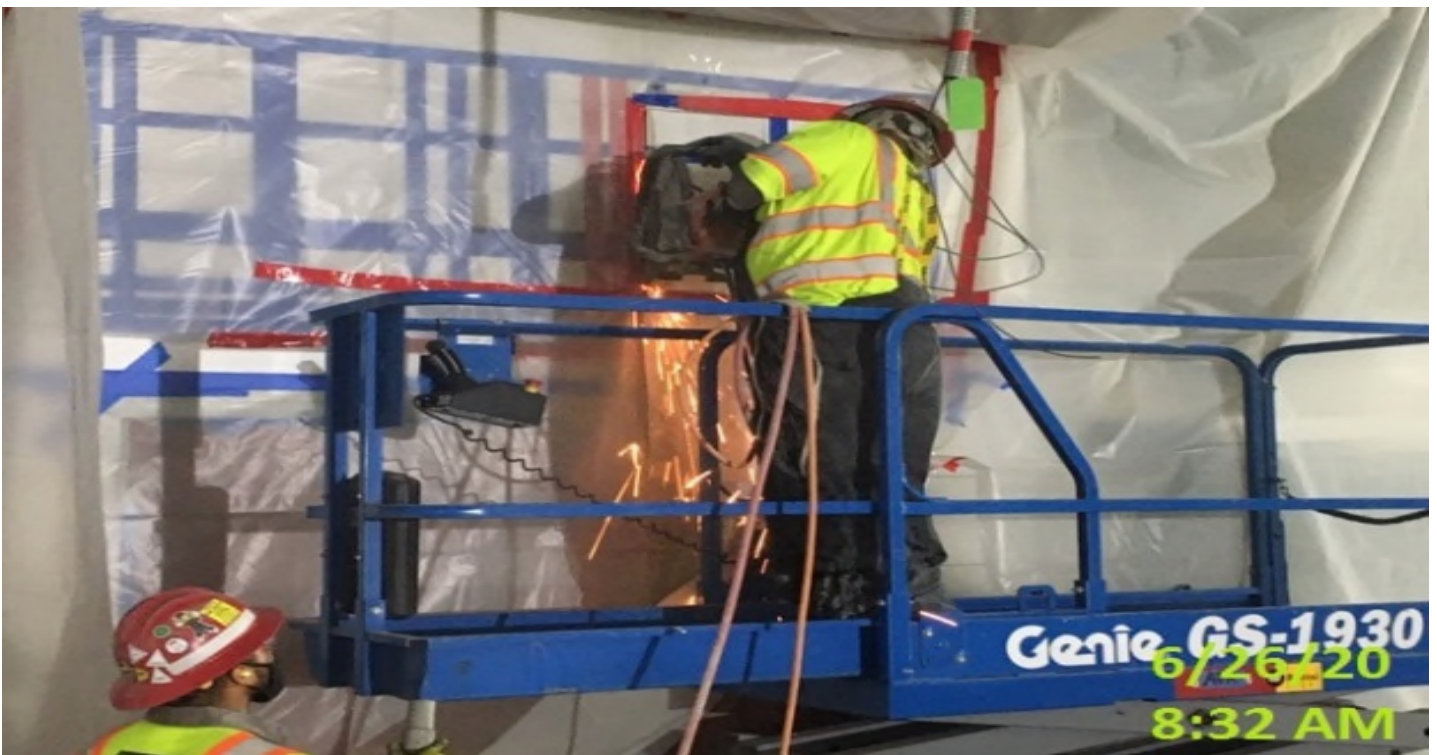
EXPO STATION- WSCC ironworkers using chain fall rigging to set in place and anchor hoist beam.
