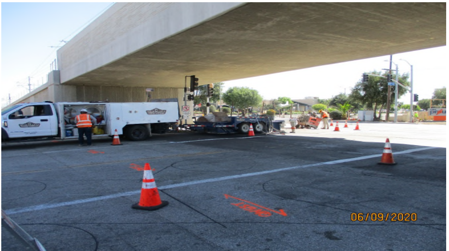
111th Street- Saw cutting the existing roadway Ac for potholing at 111th street. Facing NW.
