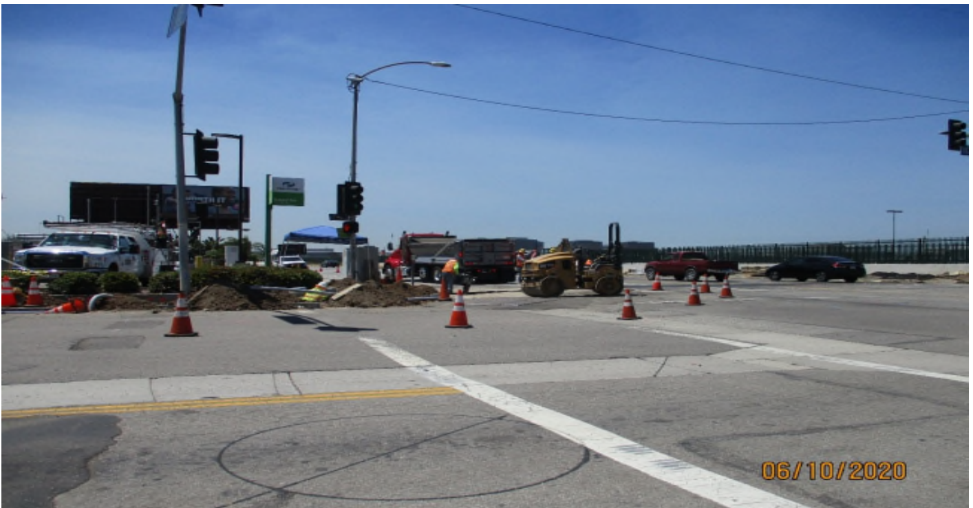
AVIATION/CENTURY- Placing and compacting AC for the traffic signal trench top on Aviation at 104th street. Facing south.
