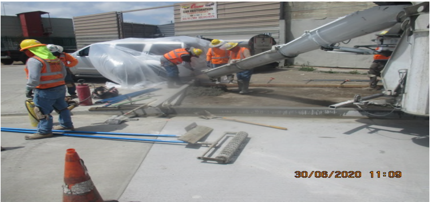
UG3 – Continue installing block-out forms and placing concrete for new sidewalk panels for the Victoria Cul-de-sac radius. 6/30/20
