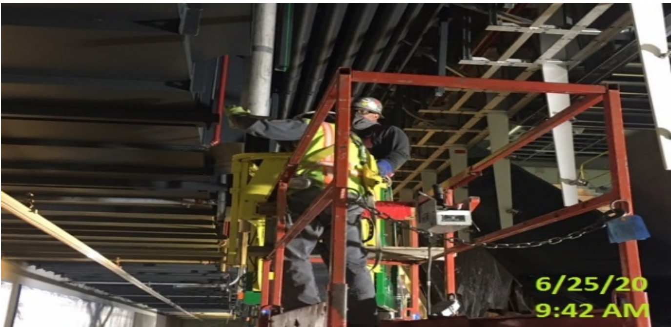
EXPO STATION – Continue welding and plumbing southbound edge light support poles along the platform level.
