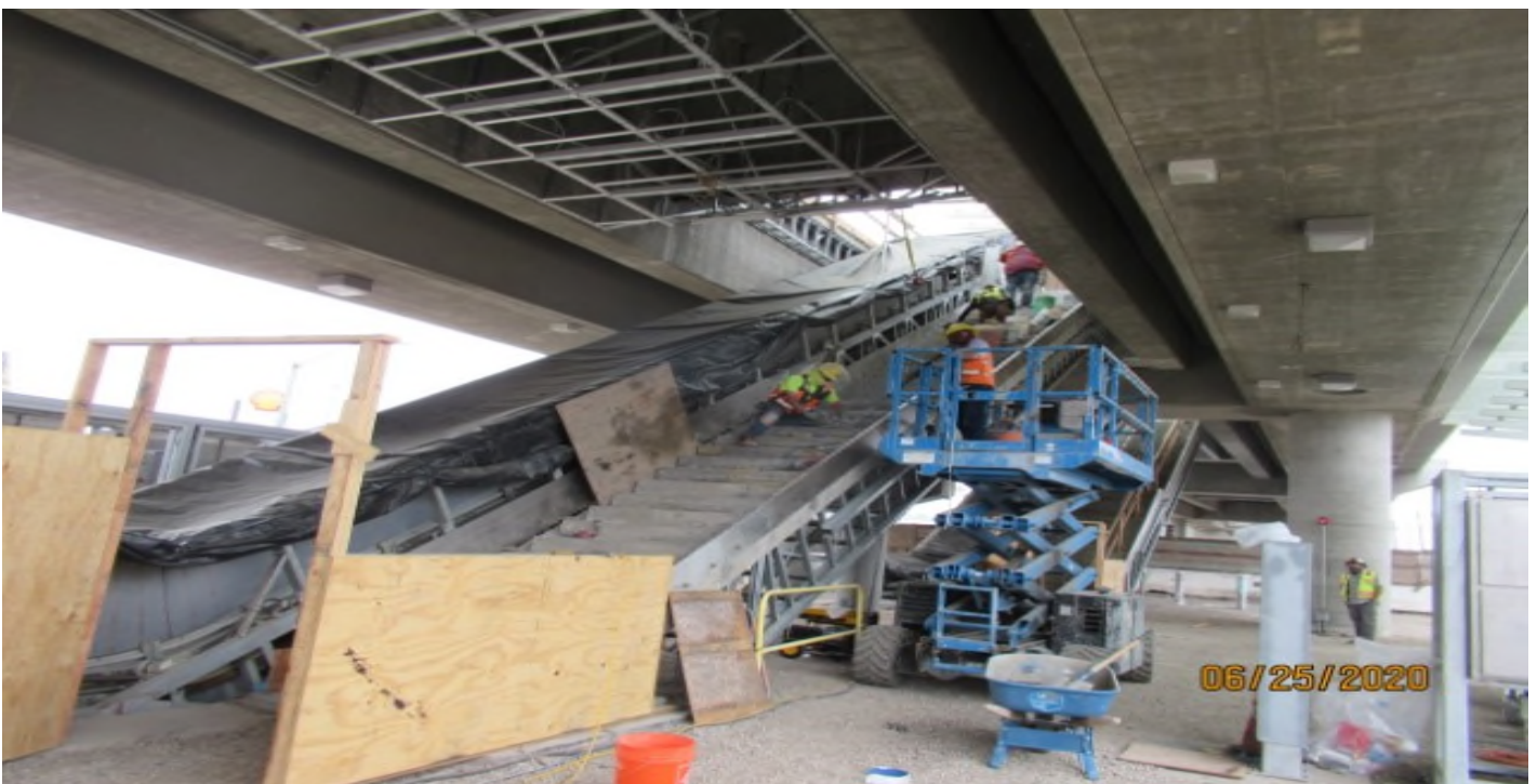
AVIATION/CENTURY- Carrera Marble & WSCC working together on stairway #1 at Century/Aviation plaza (looking south)
