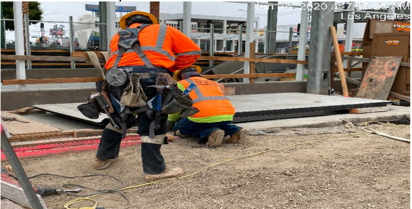
LEIMERT PARK STATION – Installing hatches to Emergency Exit Stair #2 at the plaza level.
