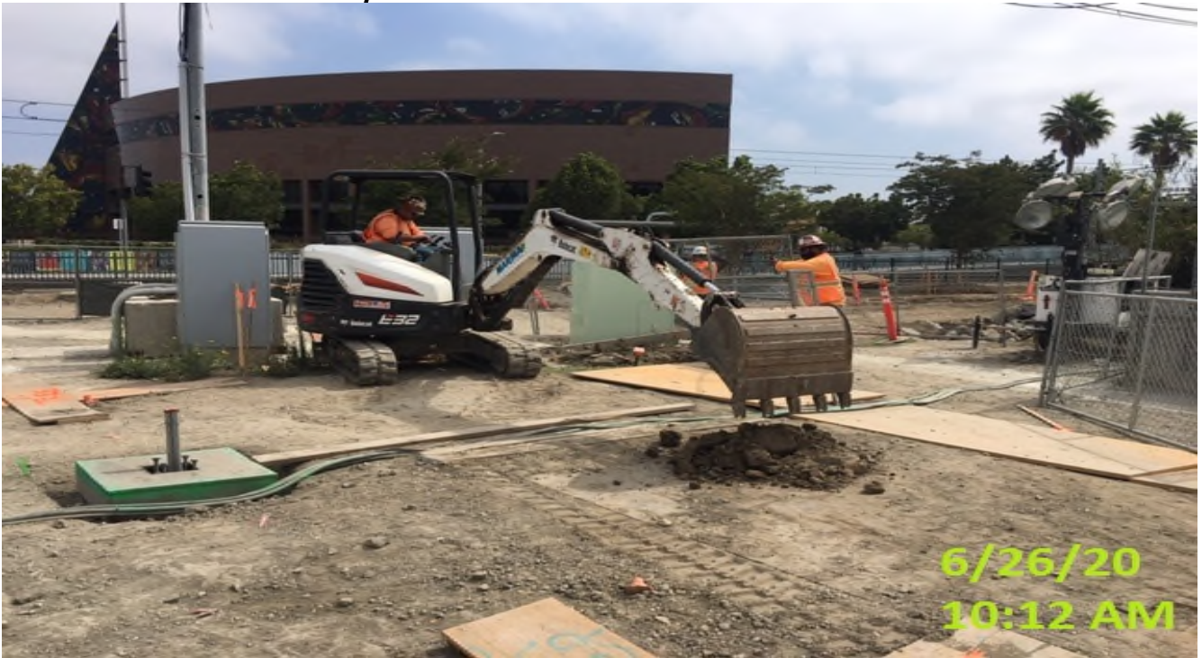
EXPO STATION – Excavating wells for palm tree installation throughout the plaza level.
