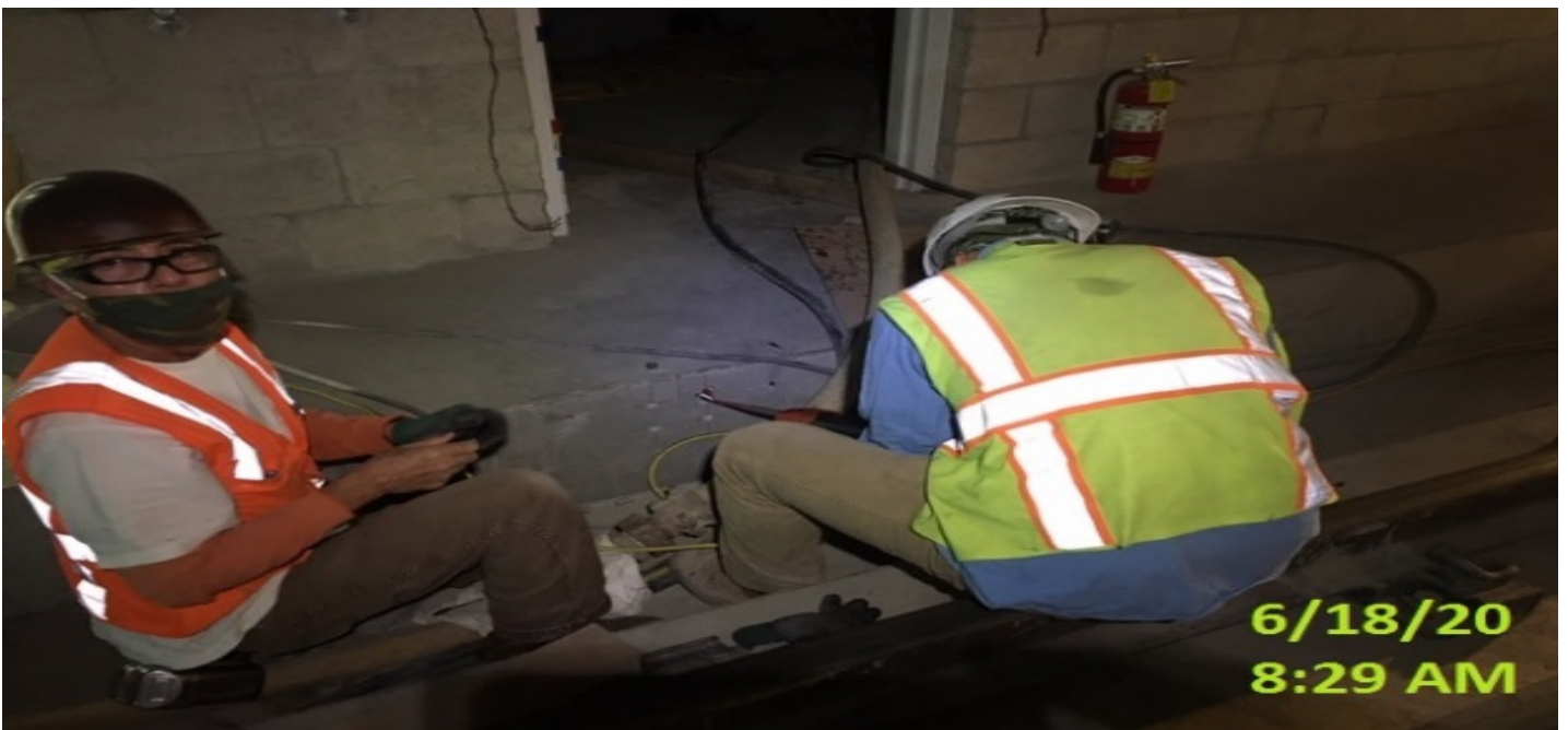
LEIMERT PARK STATION – Continue guardrail installation at the north and southbound walkways of the north end platform level.
