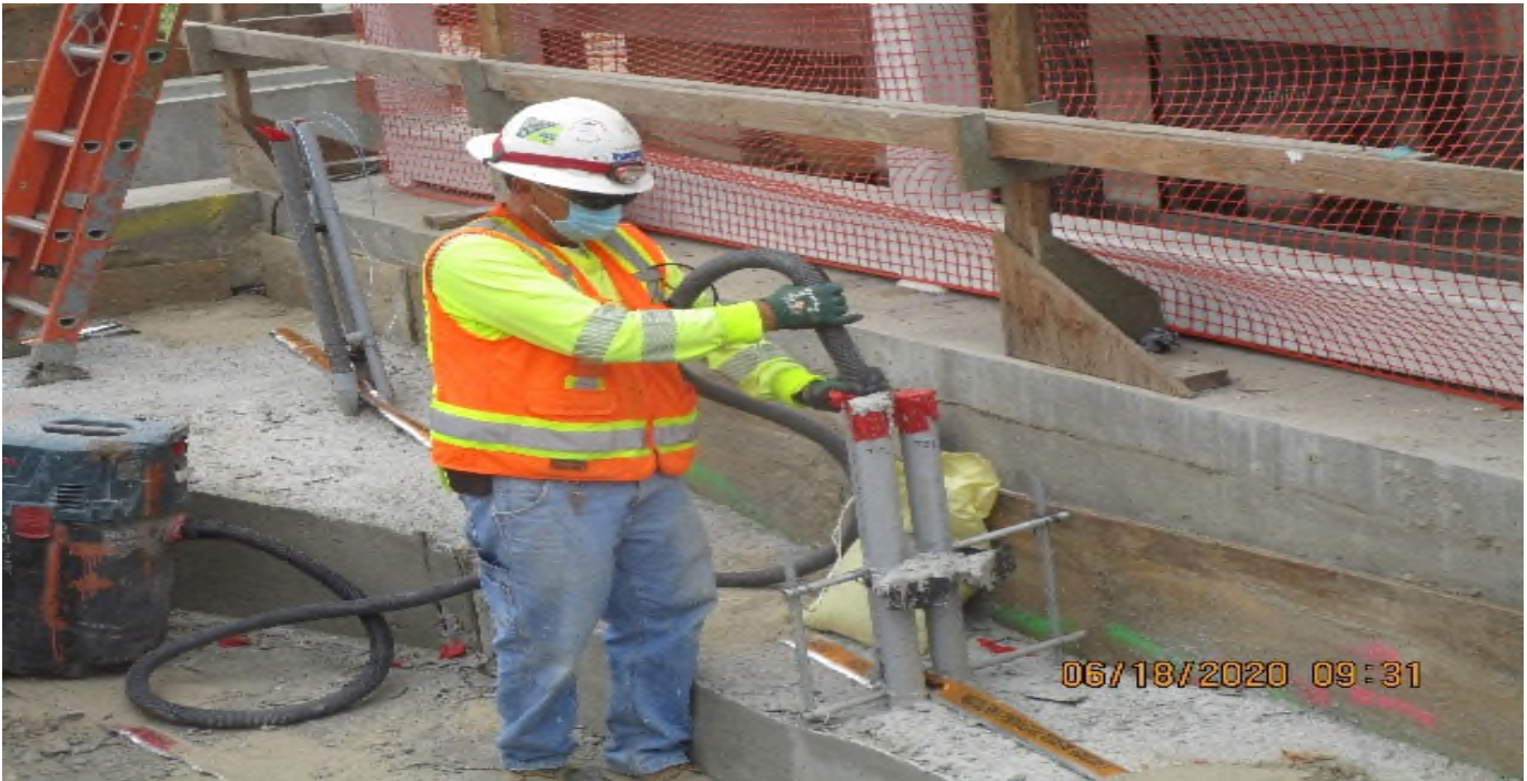
LEIMERT PARK STATION – Continue underground conduit installation for landscape lighting and utilities at the plaza level.
