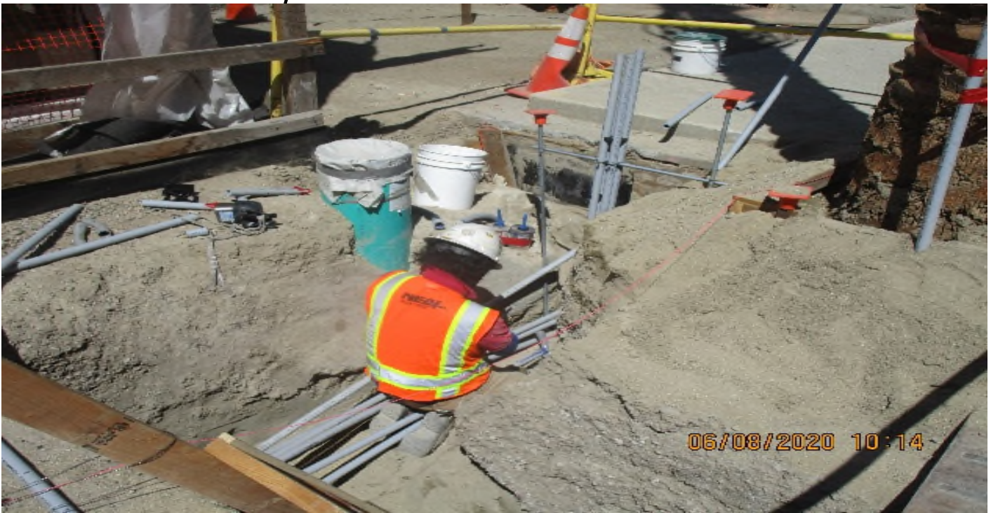
LEIMERT PARK STATION – Continue underground conduit installation for landscape lighting and utilities at the plaza level.
