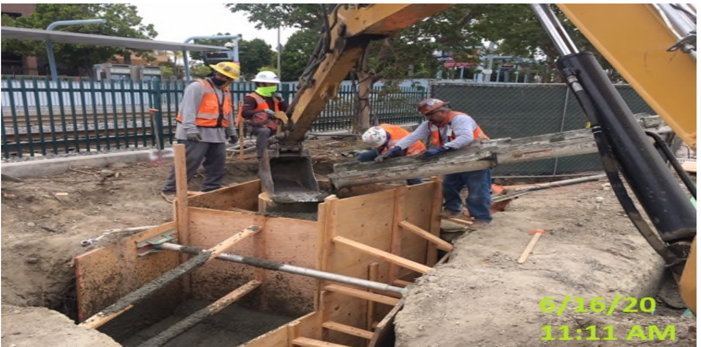
EXPO STATION – Placed concrete for manhole #1 on the northwest corner of the plaza.
