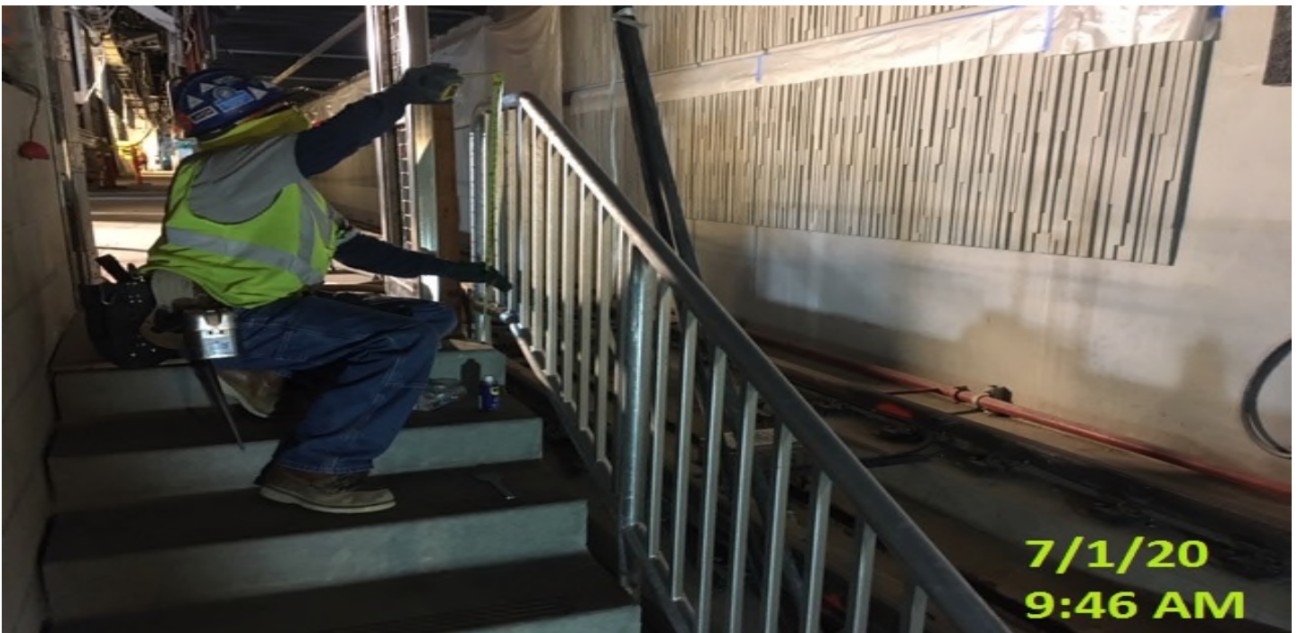
MLK STATION – Continue installing guardrails for both south and northbound tunnels at the north end invert level.
