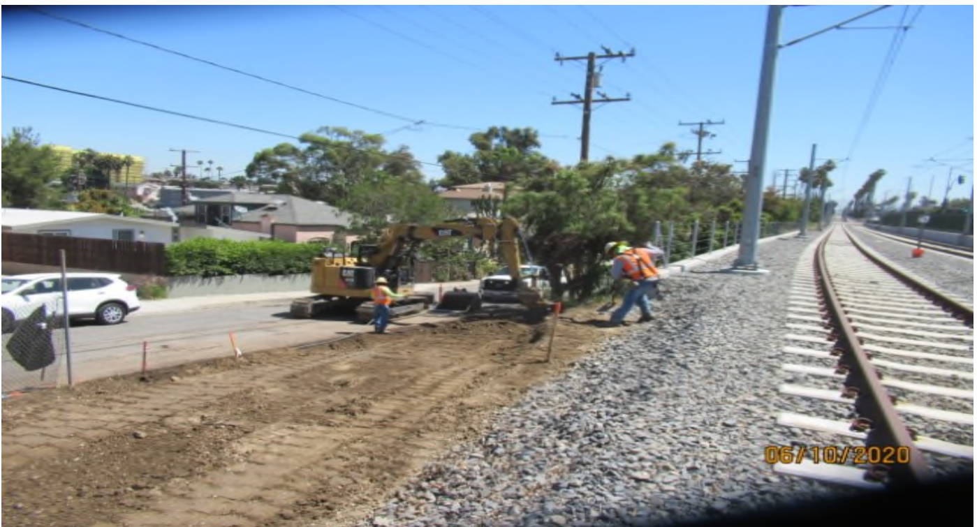
La Brea – WSCC on west side of La Brea, adding soils to slope & compacting using sheepfoot (looking north)
