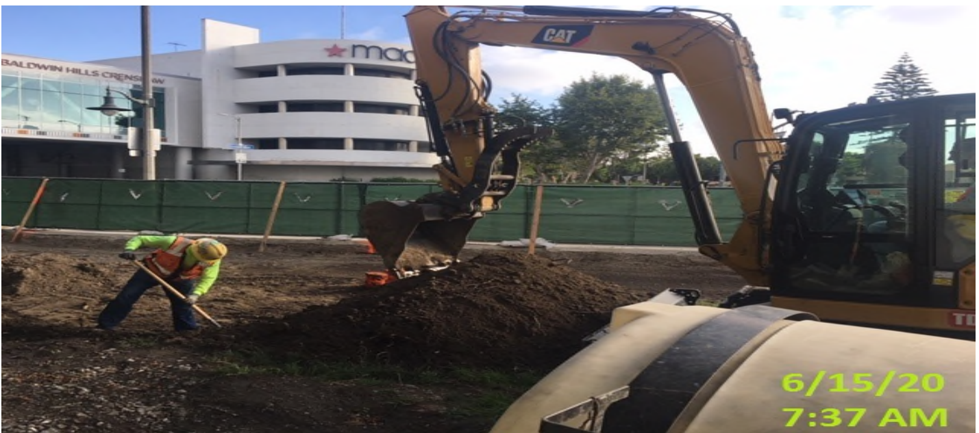
MLK - Continue excavating for upcoming paver and sidewalk installation at the north end of the plaza level.
