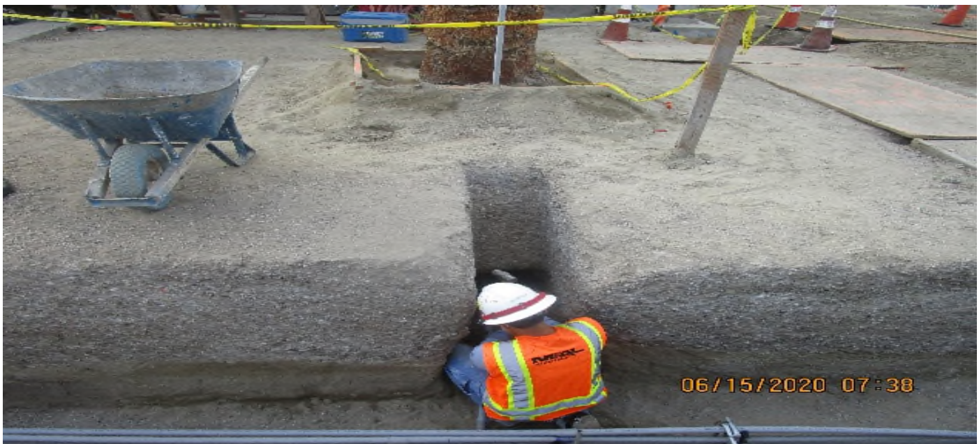
LEIMERT PARK STATION – Continue underground conduit installation for landscape lighting and utilities at the plaza level.
