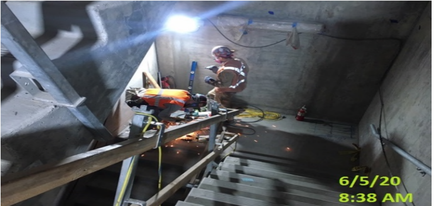
MLK STATION – Continue installing handrails at the emergency exit stairs south #2 from concourse to invert level.
