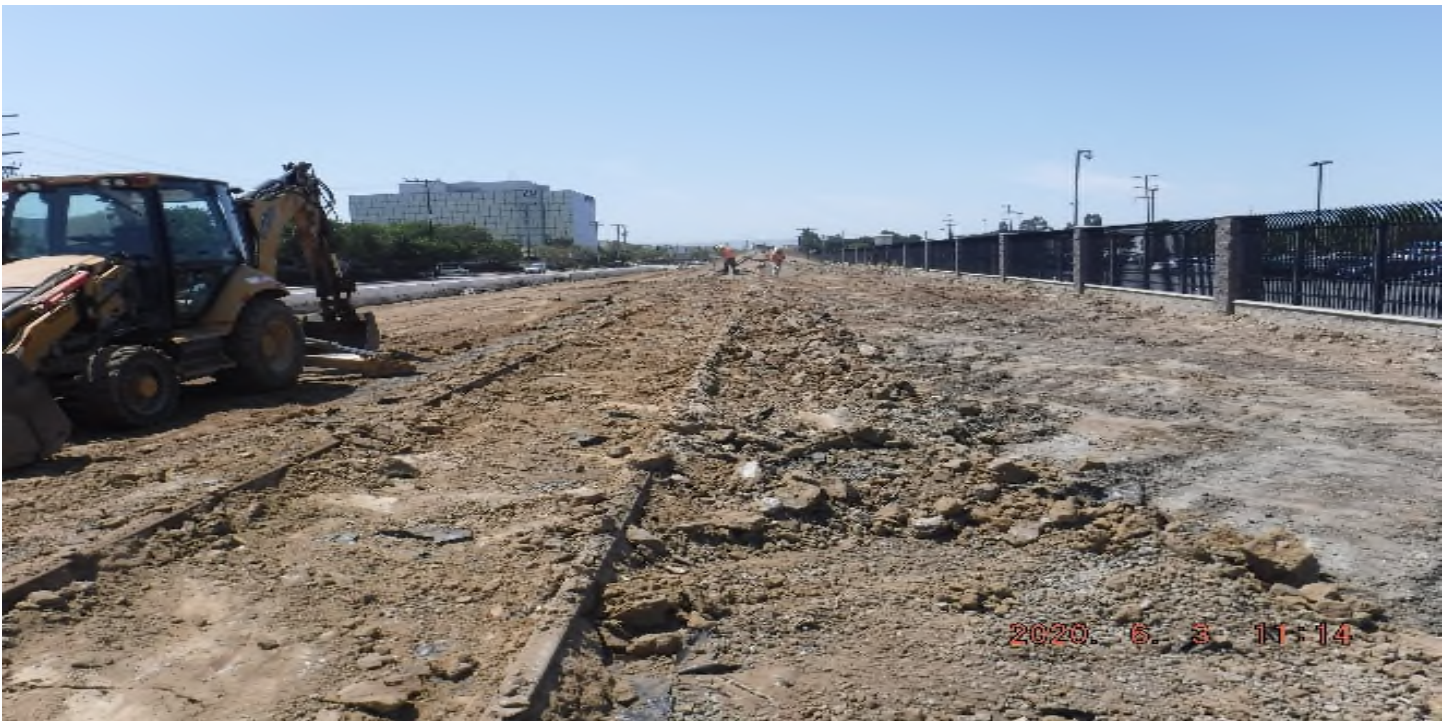
AVIATION/CENTURY- South of 124th St looking south – dirt stockpile removal from BNSF R/W and reclaim the site.
