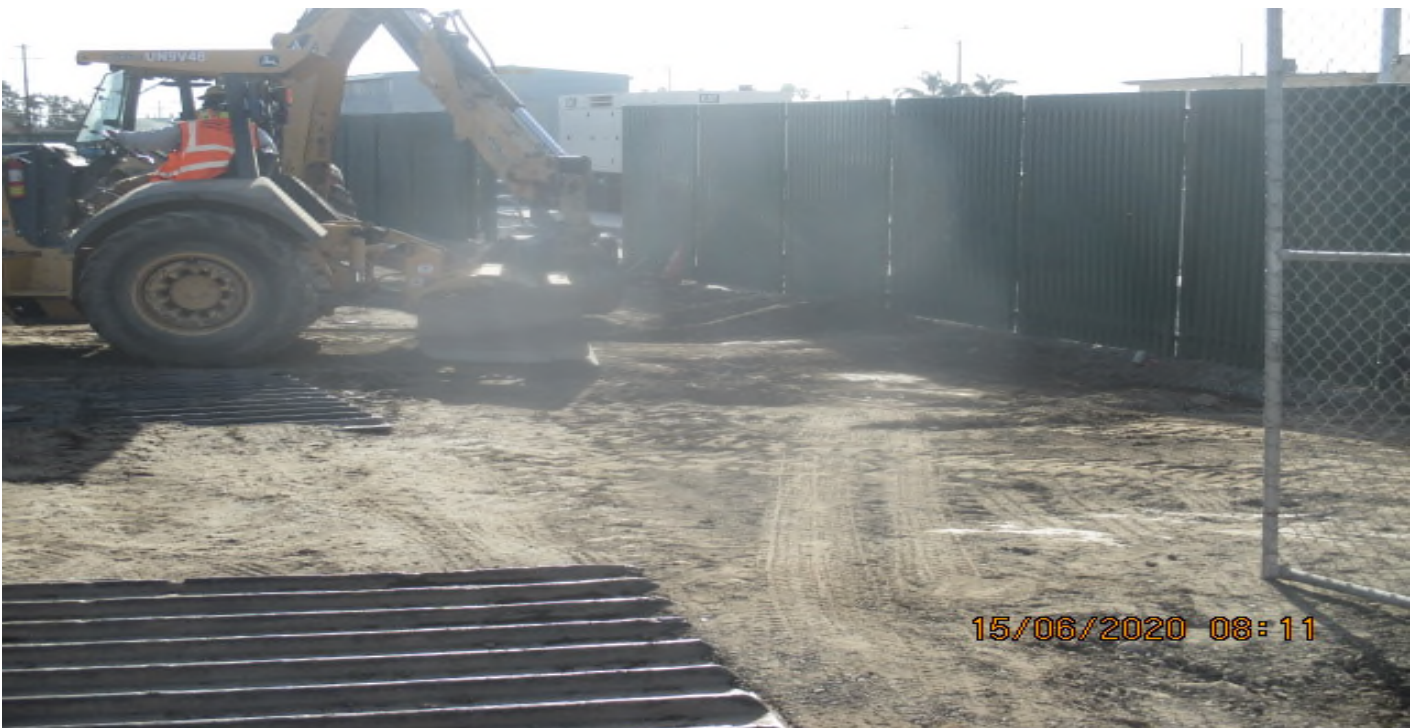
UG3 – Continue grading the north east section of Victoria Yard for upcoming pavement installation. 6/15/20
