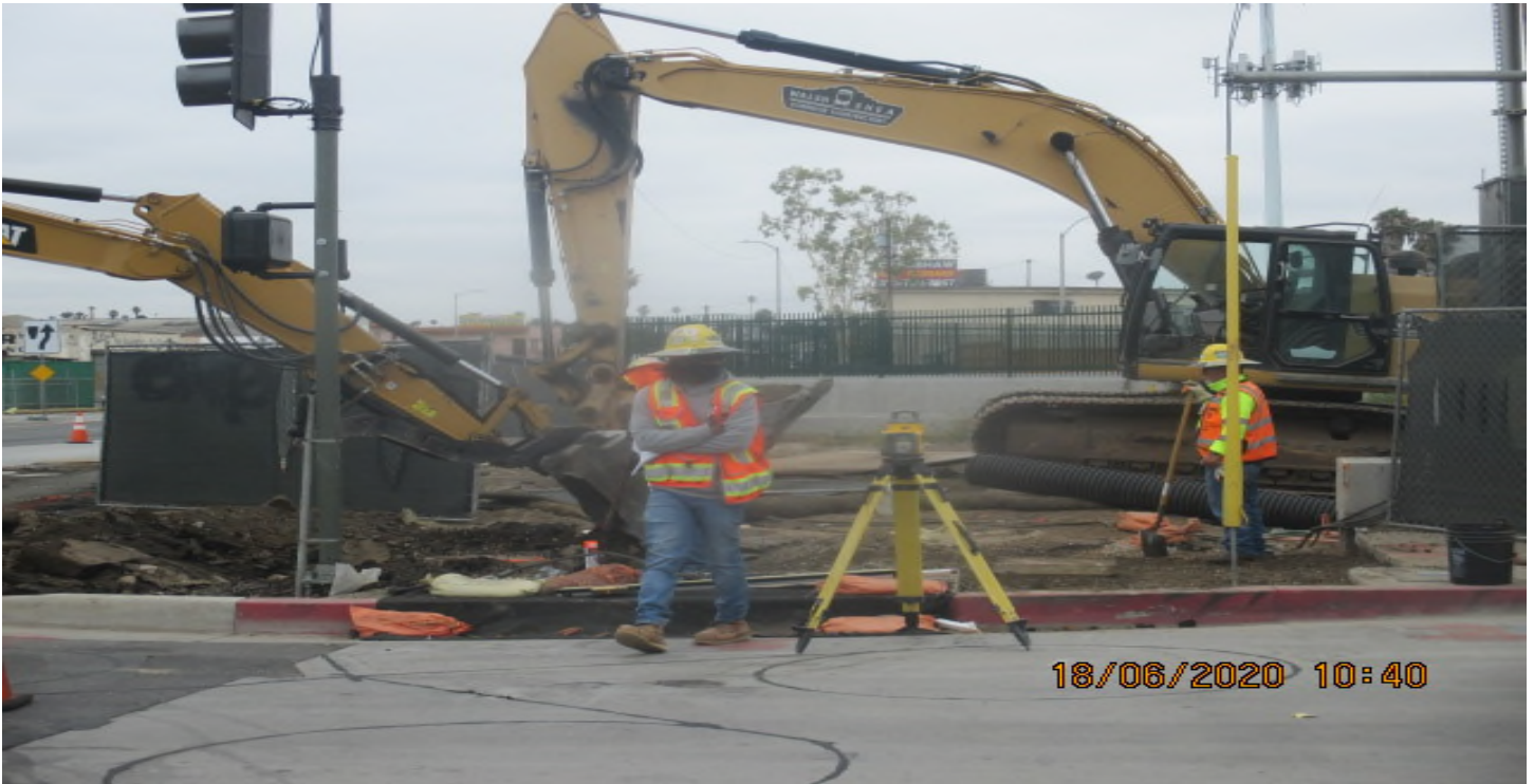
PARK MESA – Excavating/grading for new sidewalk installation on the southwest corner of 67th St & Crenshaw Blvd. 6/18/20
