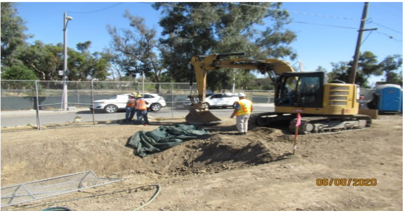
La Brea – WSCC dirt crew on west side of La Brea station, repairing temp. fence lines.
