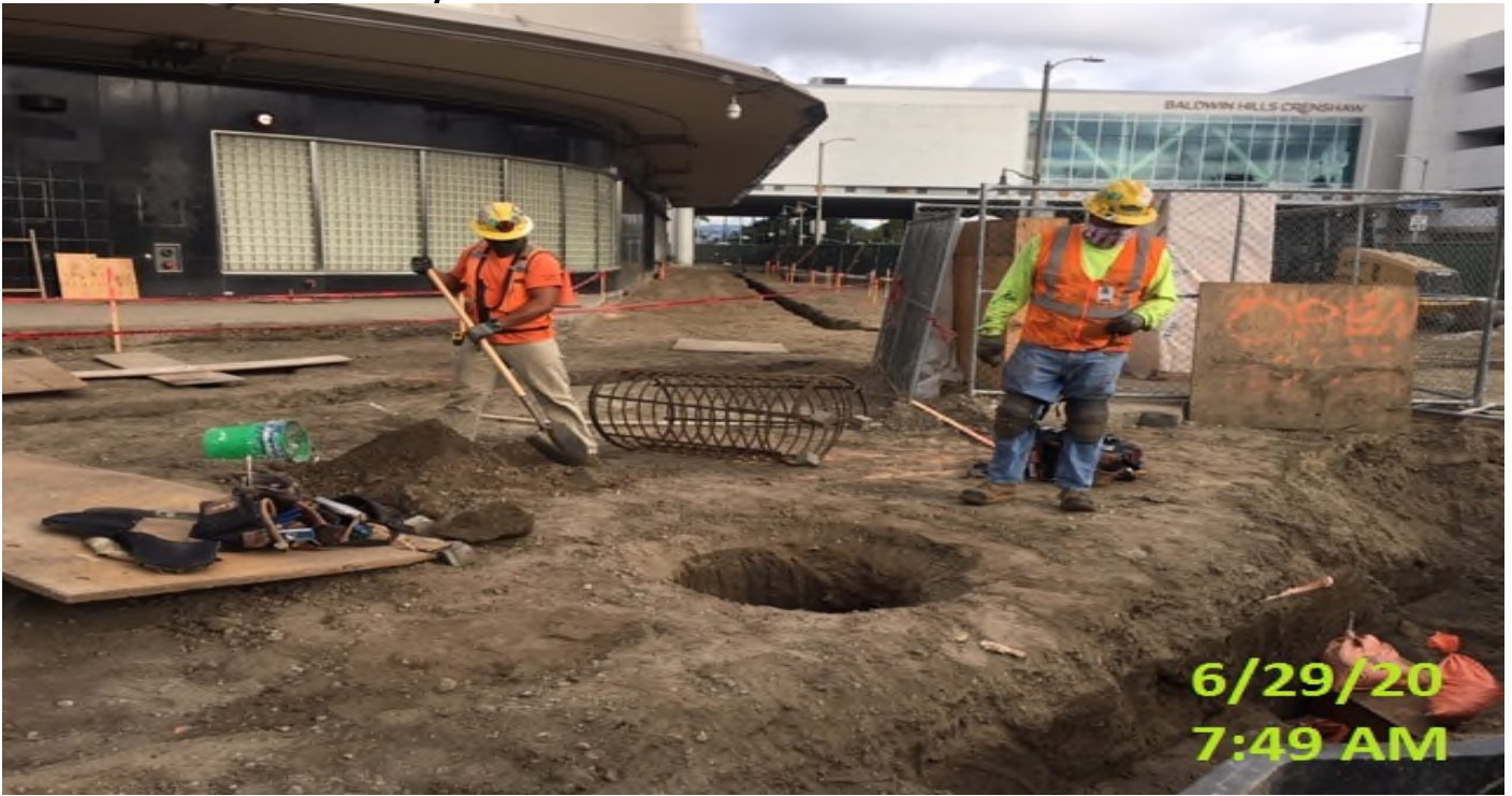
MLK STATION – Setting rebar cages for pedestrian light pole foundations throughout the plaza level.
