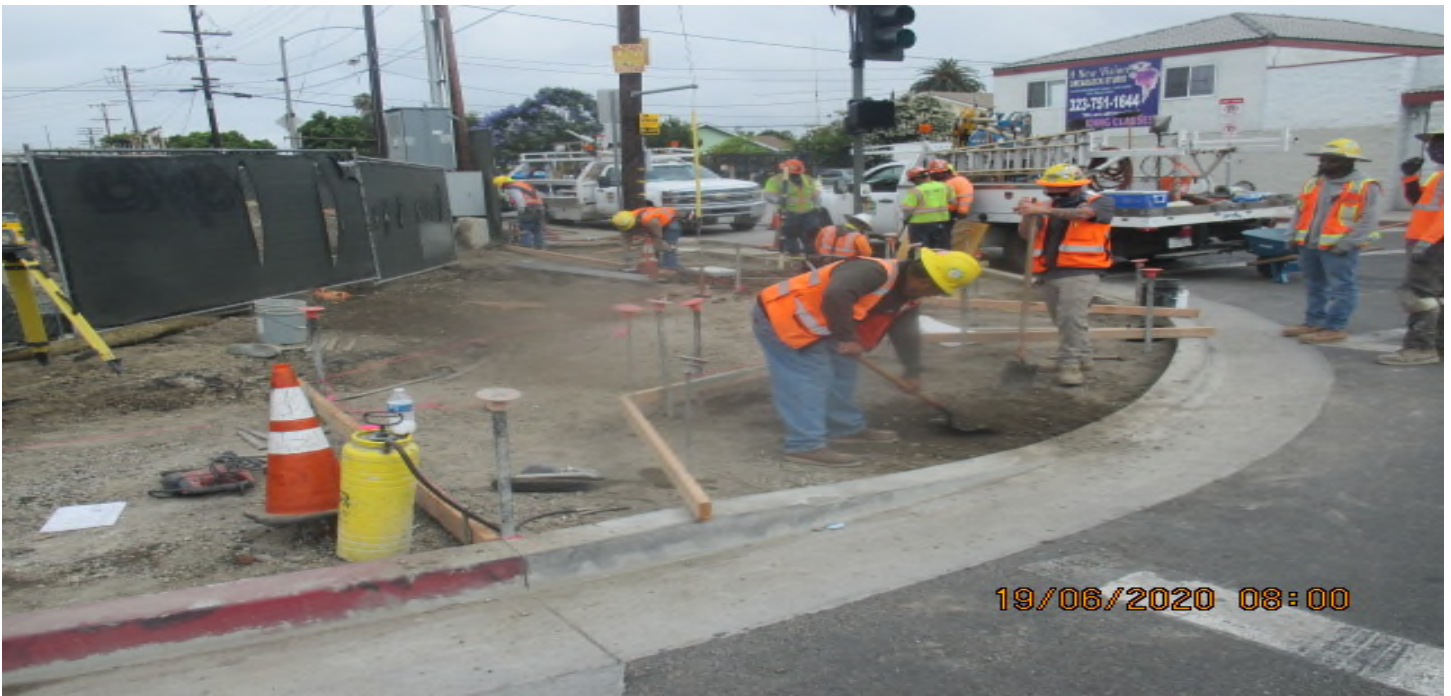
PARK MESA – Build block-out forms for ADA ramp installation and light pull boxes on the southwest corner of 67th St & Crenshaw Blvd. 6/19/20
