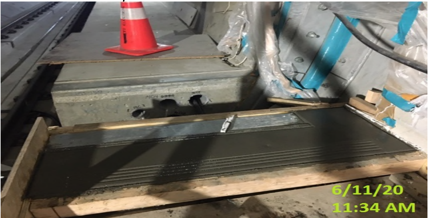
EXPO STATION – Encased embed in concrete for the stair landings of the northbound emergency walkway in the invert level.
