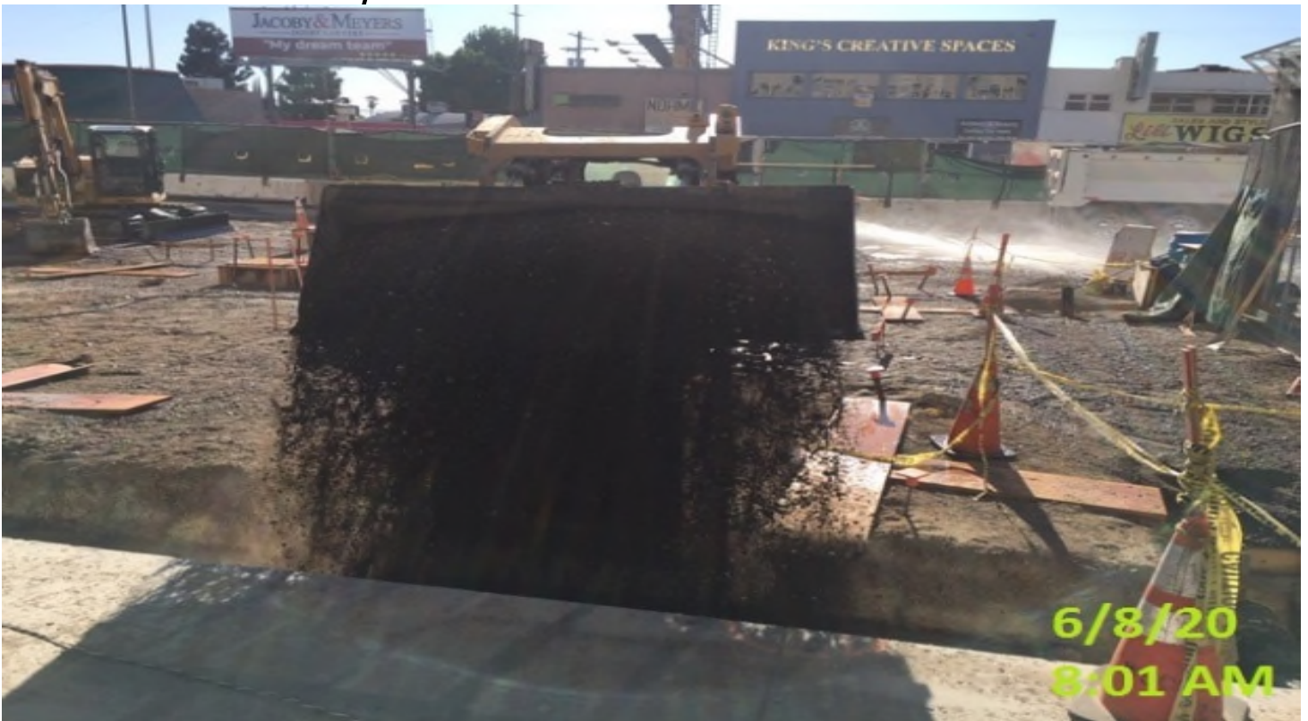
MLK STATION- WSCC crew backfilling encased 12" HDPE drain line with base grade.
