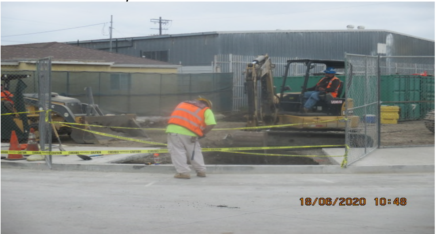
UG3 – Fine grading for tree well installation at the east side radius of the Victoria Cul-de-sac. 6/18/20
