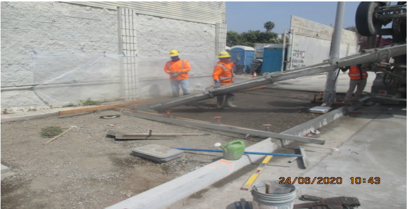
UG3 – Installing block-out forms and placing concrete for new sidewalk panels for the Victoria Cul-de-sac radius. 6/24/20
