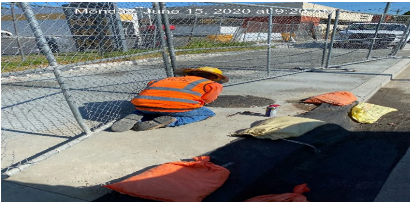
EXPO STATION – Drilling and installing bolts for manhole lid on southbound Crenshaw Blvd between Exposition Blvd and Obama Blvd.
