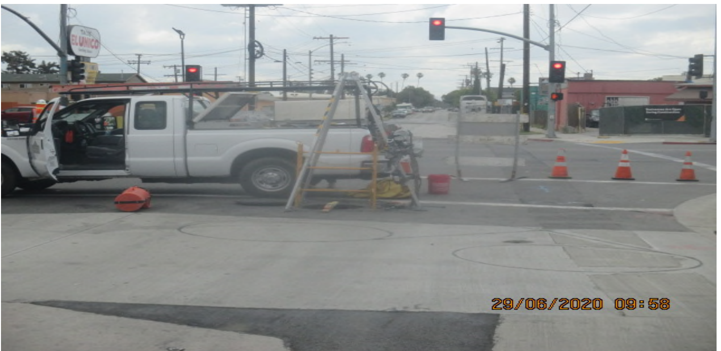
PARK MESA – Sack and patching Manhole #4 on the southwest corner of 67th St & Crenshaw Blvd. 6/29/20
