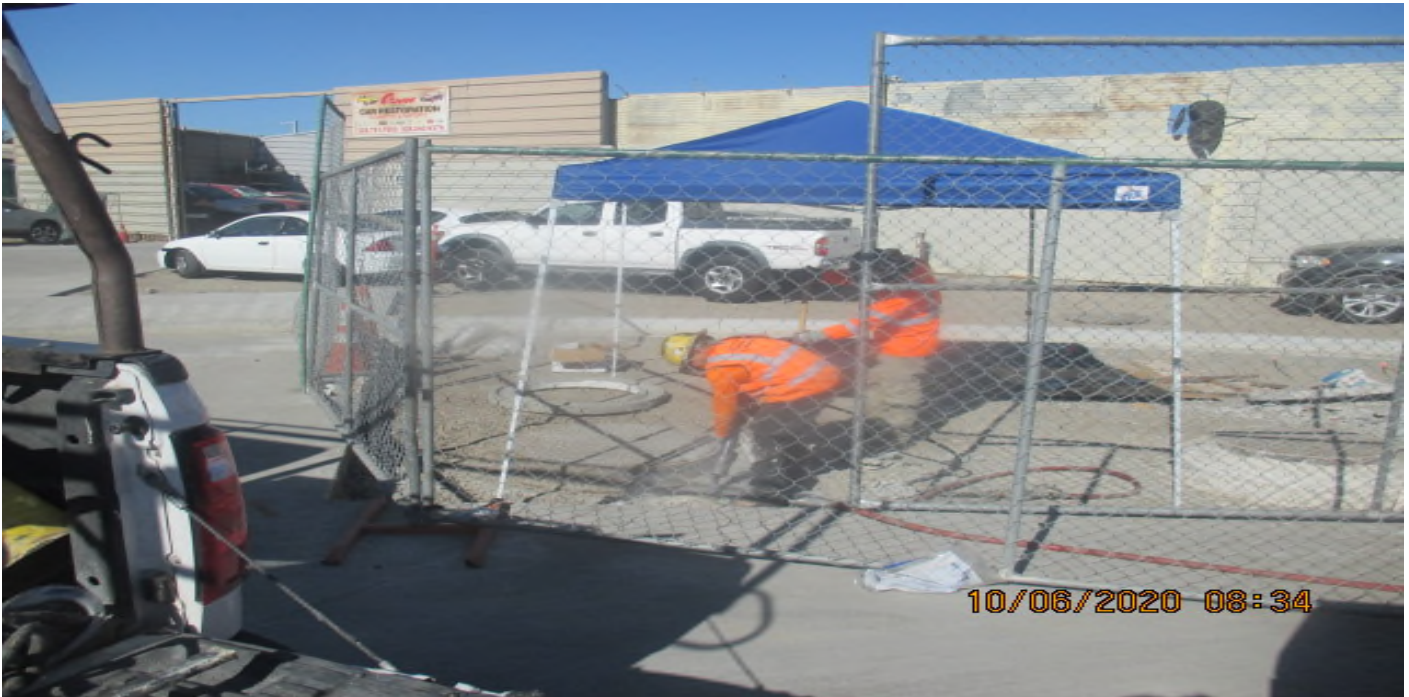
UG3 – Raising top elevation of existing manholes to road elevation at the Victoria Cul-de-sac. 6/10/20
