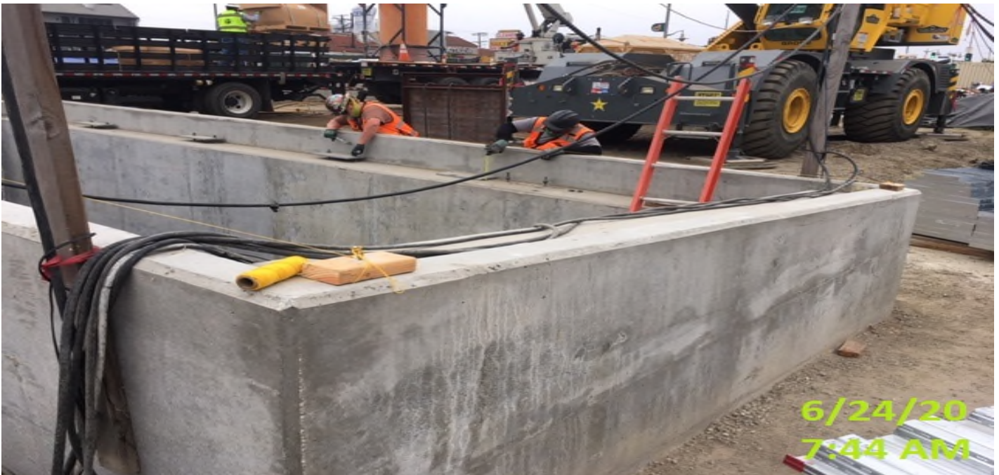
MLK STATION – Installing steel grating for the south air exhaust vent shaft at the plaza level.
