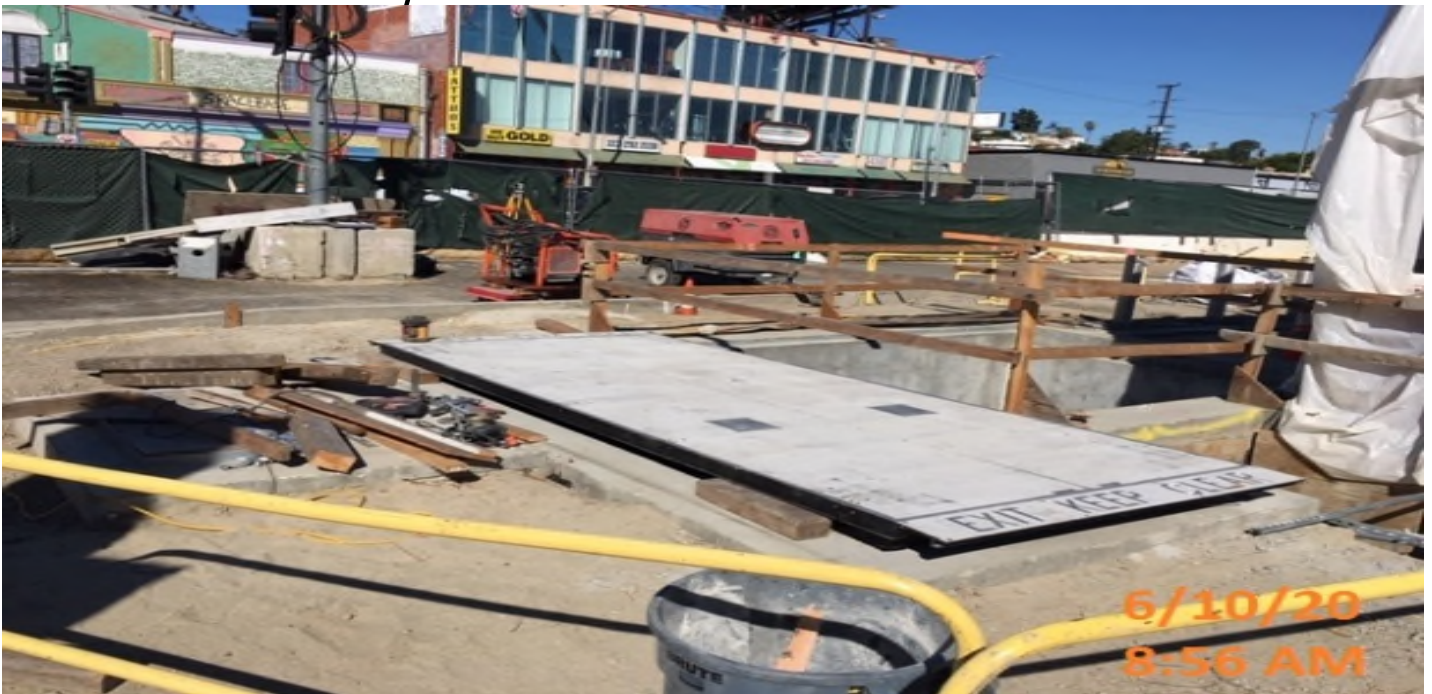
LEIMERT PARK STATION – Installed hatch for the Emergency Exit Stair 1 at the plaza level.
