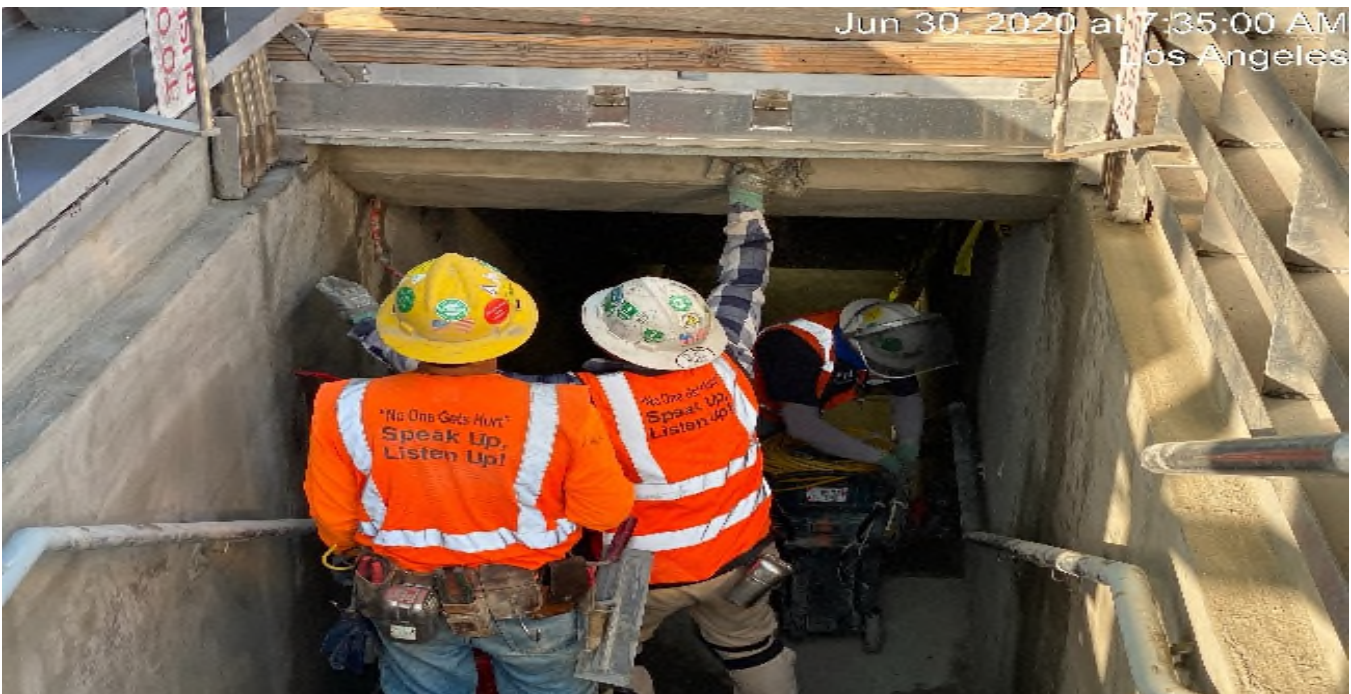
LEIMERT PARK STATION – Sack and patching the walls of Emergency Exit Stair 2 at the plaza level.
