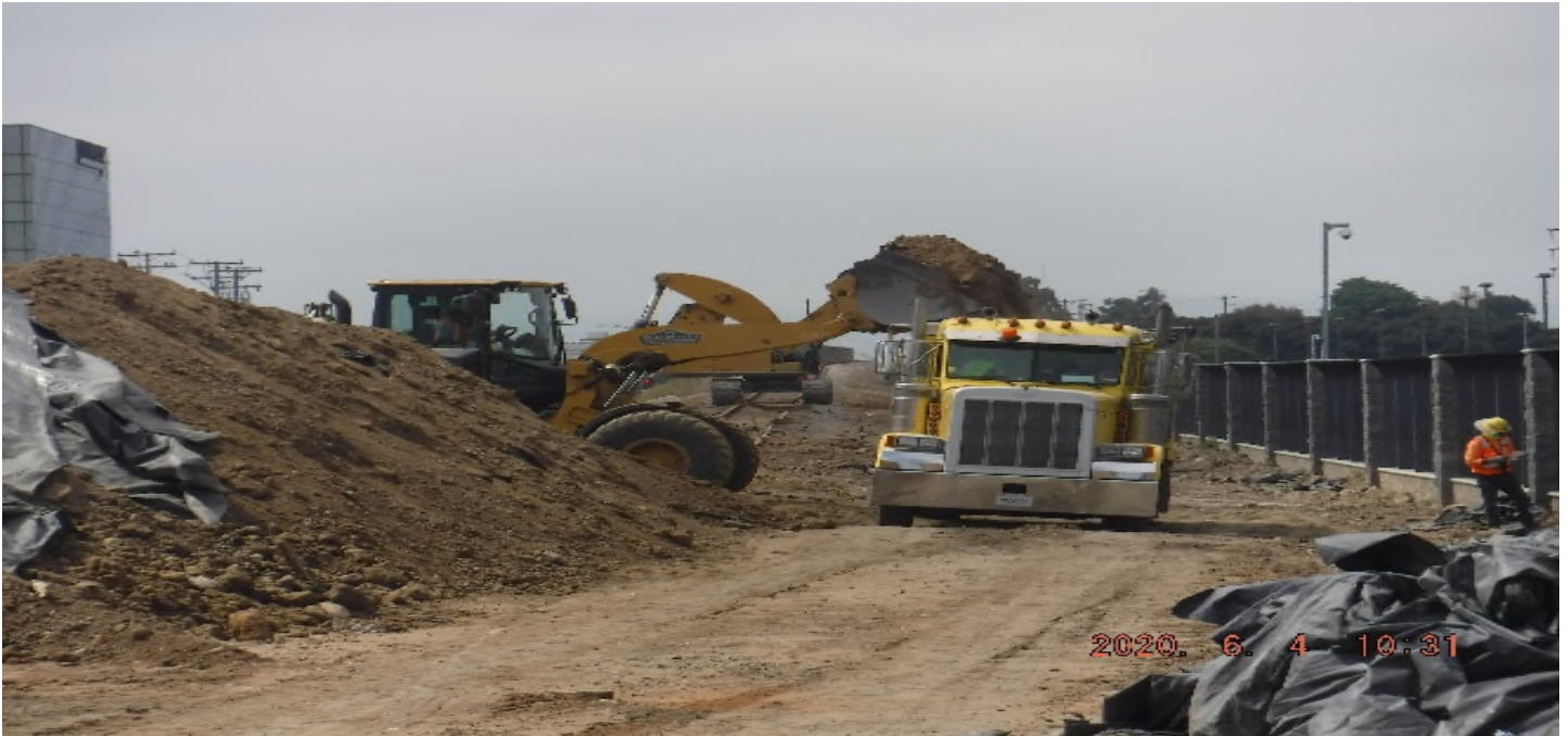
AVIATION/CENTURY- South of 124th St looking south – dirt stockpile removal from BNSF R/W and reclaim the site.
