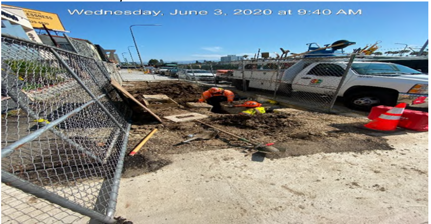
LEIMERT PARK STATION – Excavating for the installation of a street light foundation on southbound Crenshaw Blvd between 48th St and Brynhurst Ave.
