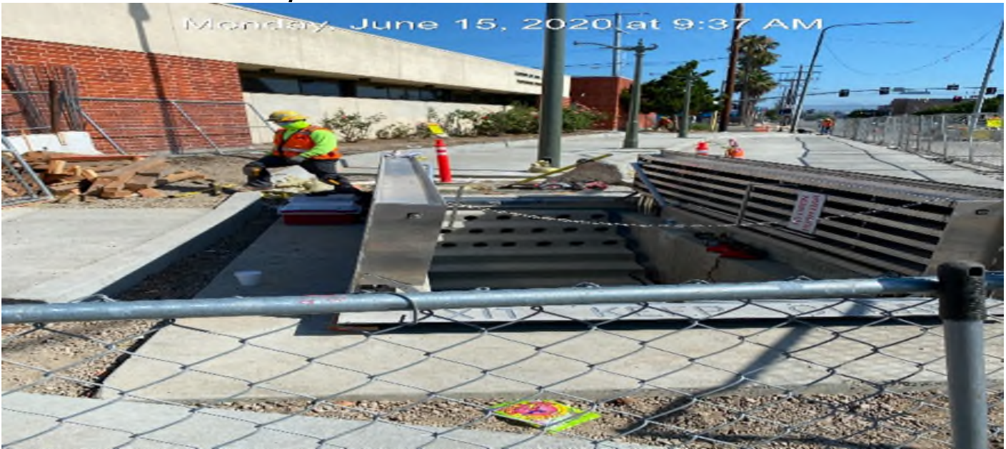
EXPO STATION – Installing hatch for North Emergency Exit Stair #2 on southbound Crenshaw Blvd between Exposition Blvd and Obama Blvd.
