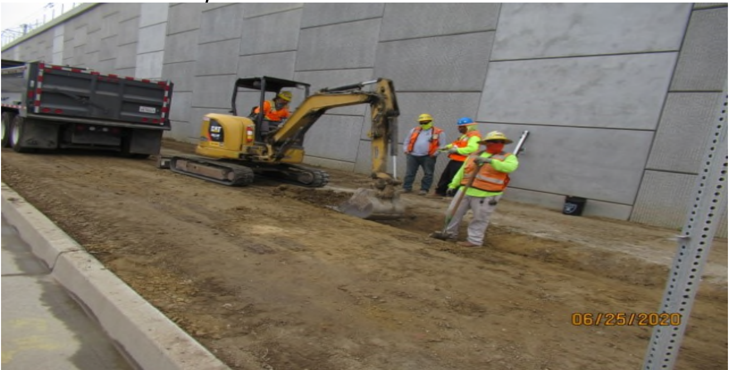
AVIATION/CENTURY- WSCC grading V-ditch along RW#60 Aviation Blvd. in Segment A using mini Excavator & 5-yard dump truck (looking southwest)
