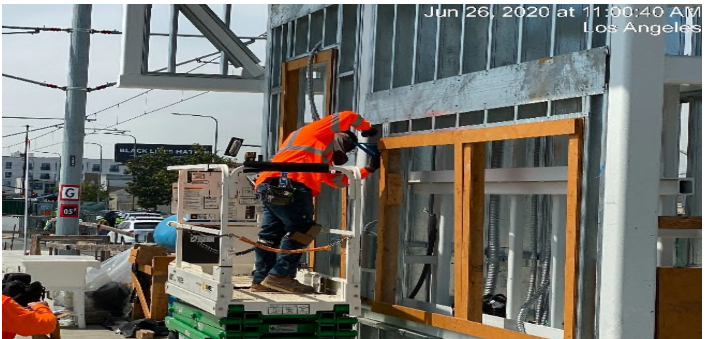
Hyde Park Station – Began layout for the upcoming ticket vending machine installation at the platform.
