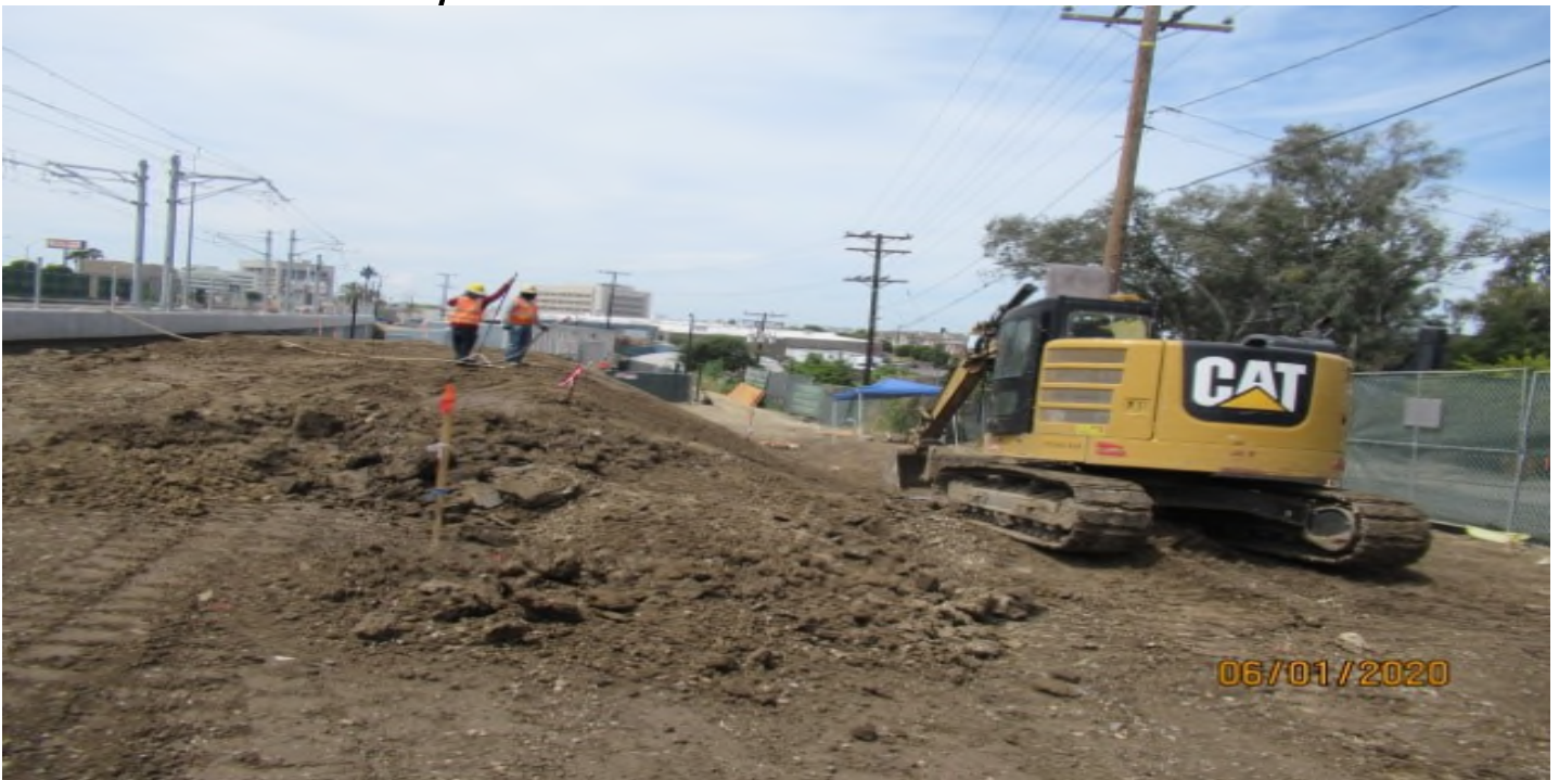
La Brea – WSCC civil dirt crew installing V-ditch, west side at La Brea (looking south)
