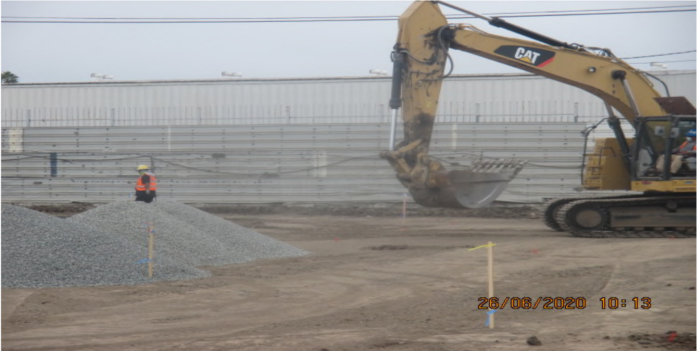
UG3 – Continue excavating/grading and stockpiling granite base rocks for upcoming placement at Victoria Yard. 6/26/20
