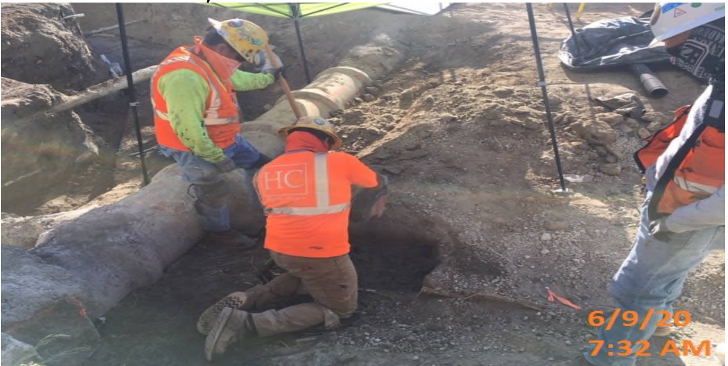
MLK Station - Excavating for pedestrian light pole foundations at the northwest side of the plaza level.
