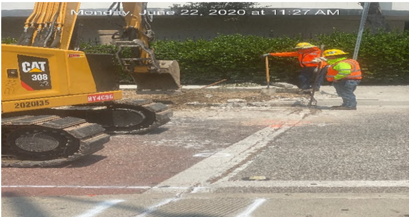
MLK STATION – Excavating/demolishing for new ADA ramp and sidewalk installation on the northwest corner of MLK Blvd and Crenshaw Blvd.
