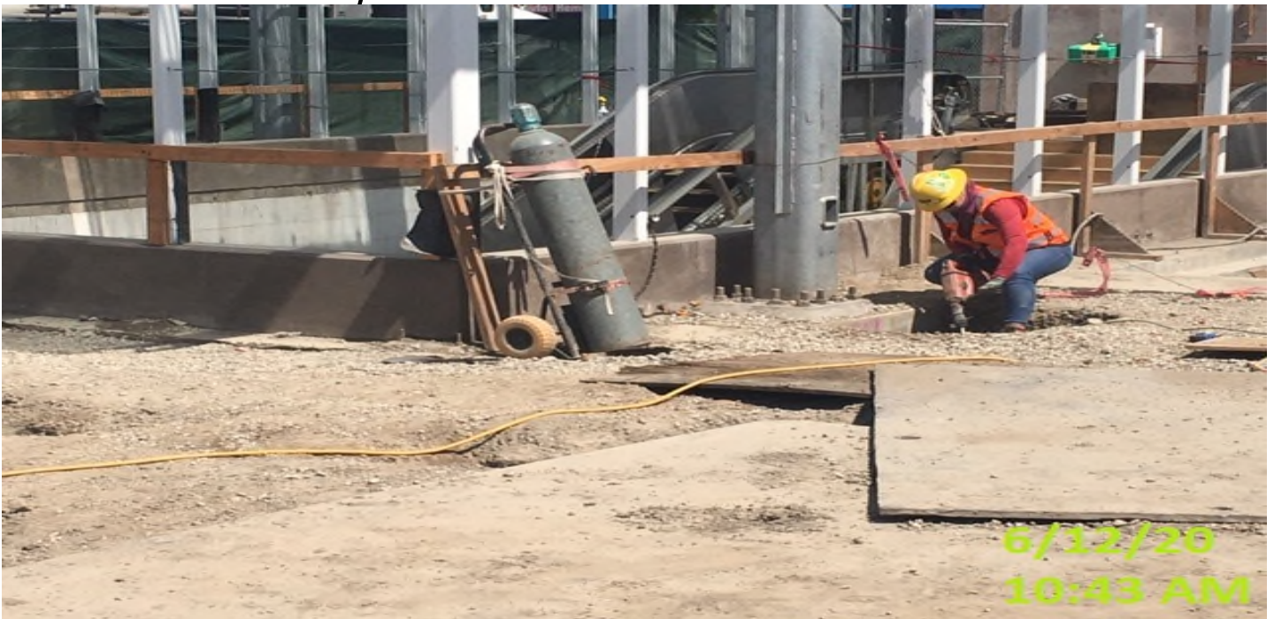
EXPO STATION- WSCC crew hand digging adjacent to canopy footings for plaza lighting stubbing.
