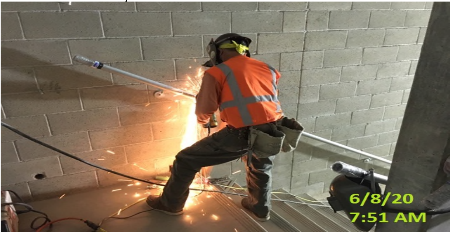
MLK STATION – Continue installing handrails at the emergency exit stairs south #2 from concourse to invert level.
