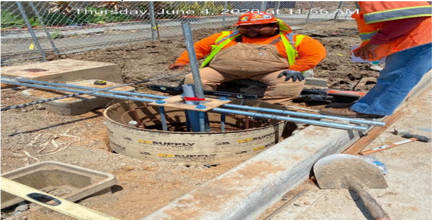
LEIMERT PARK STATION – Installing street light foundation on southbound Crenshaw Blvd between 48th St and Brynhurst Ave.
