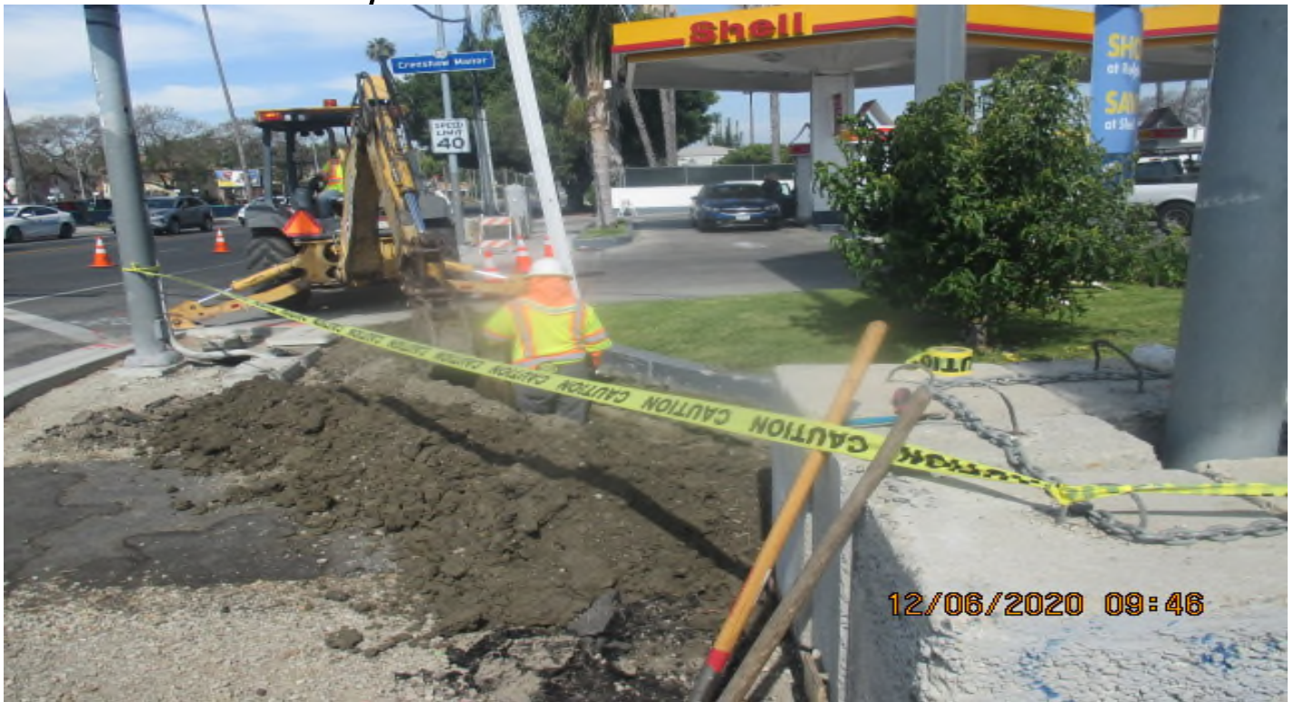
EXPO STATION – Installing conduit to supply power for the street light pole on the northwest corner of Obama Blvd and Crenshaw Blvd. 6/12/20
