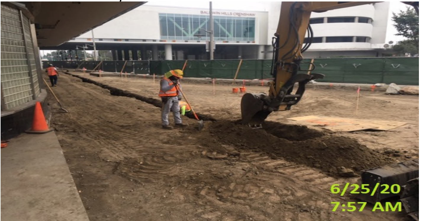
MLK STATION –Continue excavating/trenching for underground landscaping conduit installation at the west side of the plaza level.
