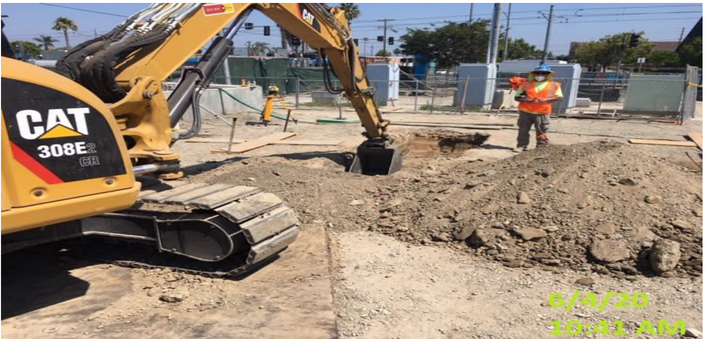
EXPO STATION – Continue excavating/trenching for map case foundation footing at the plaza.
