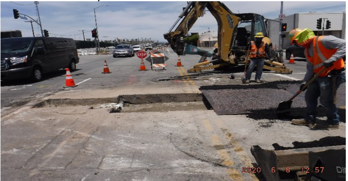
AVIATION/CENTURY- STA 55+00 at Aviation Blvd NB , 104th St looking north – trench work for traffic conduits in progress.
