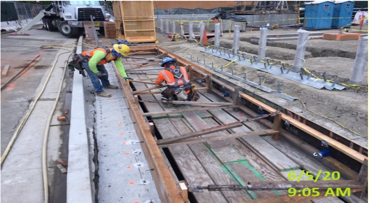
MLK STATION- WSCC crew building formwork for air exhaust shaft, per NCR.
