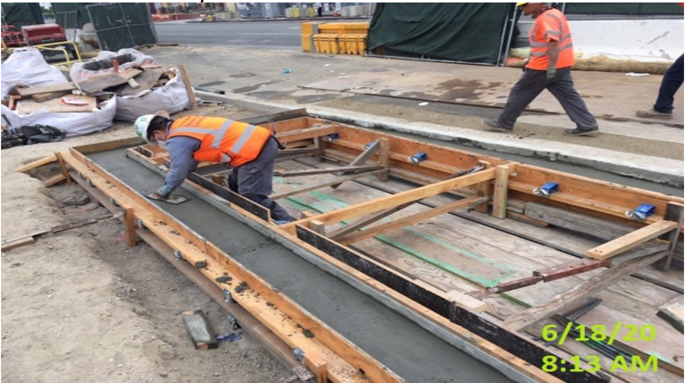
LEIMERT PARK STATION – Placing concrete for the air exhaust shaft at the plaza level.
