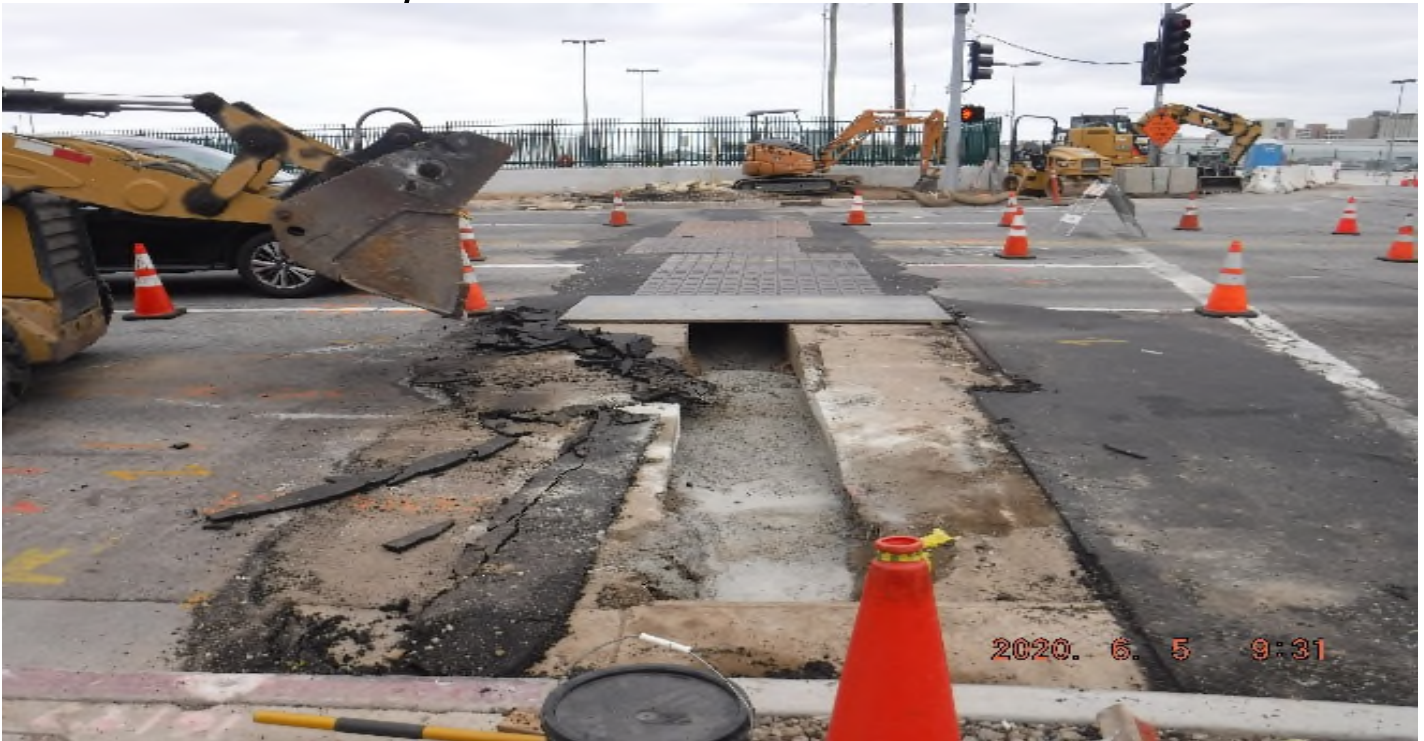
AVIATION/CENTURY- STA 55+00 at Aviation Blvd NB , 104th St looking west – slurry placed in trench work for traffic conduits.
