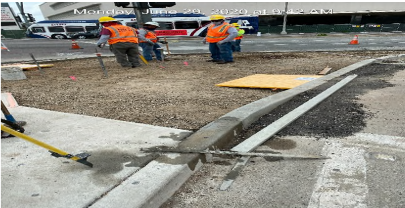
MLK STATION – Continue building formwork for new ADA ramp and curb/gutter installation on the west median corner of MLK Blvd and Crenshaw Blvd.
