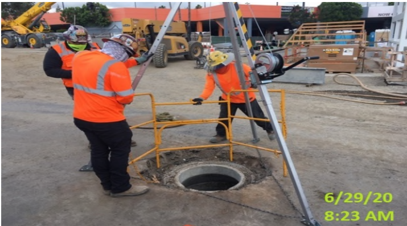
MLK STATION – Chipping and patching inside Man Hole #15 at the plaza level.
