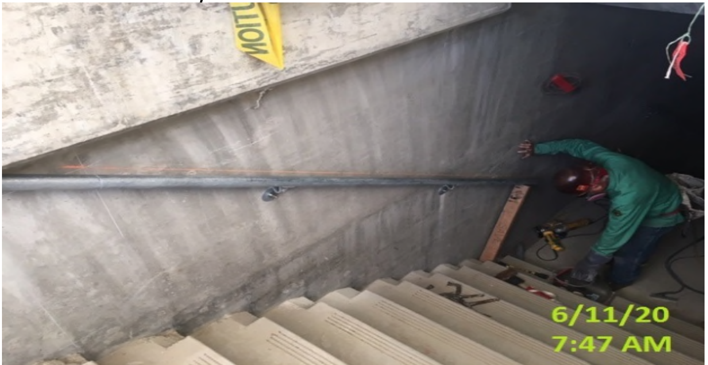
MLK STATION – Continue installing handrails at the emergency exit stairs south #2 from concourse to invert level.
