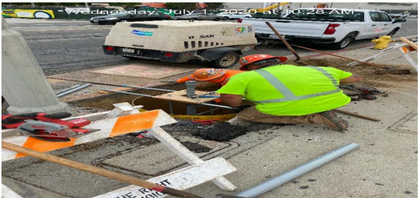
MLK STATION – Installing pedestrian signal head foundations on Crenshaw Blvd between Stocker St and MLK Blvd.
