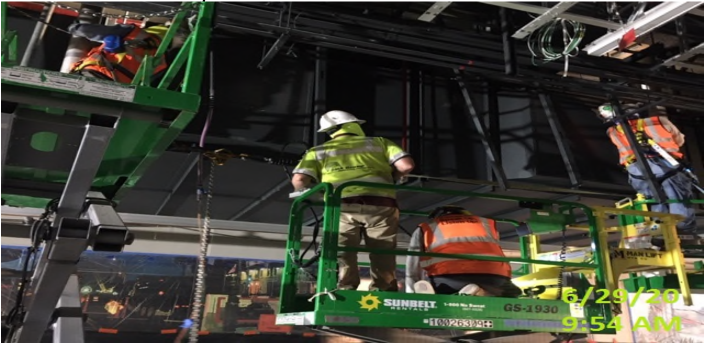
EXPO STATION- WSCC crew performing pull tests on edge lighting down stand embed plates.
