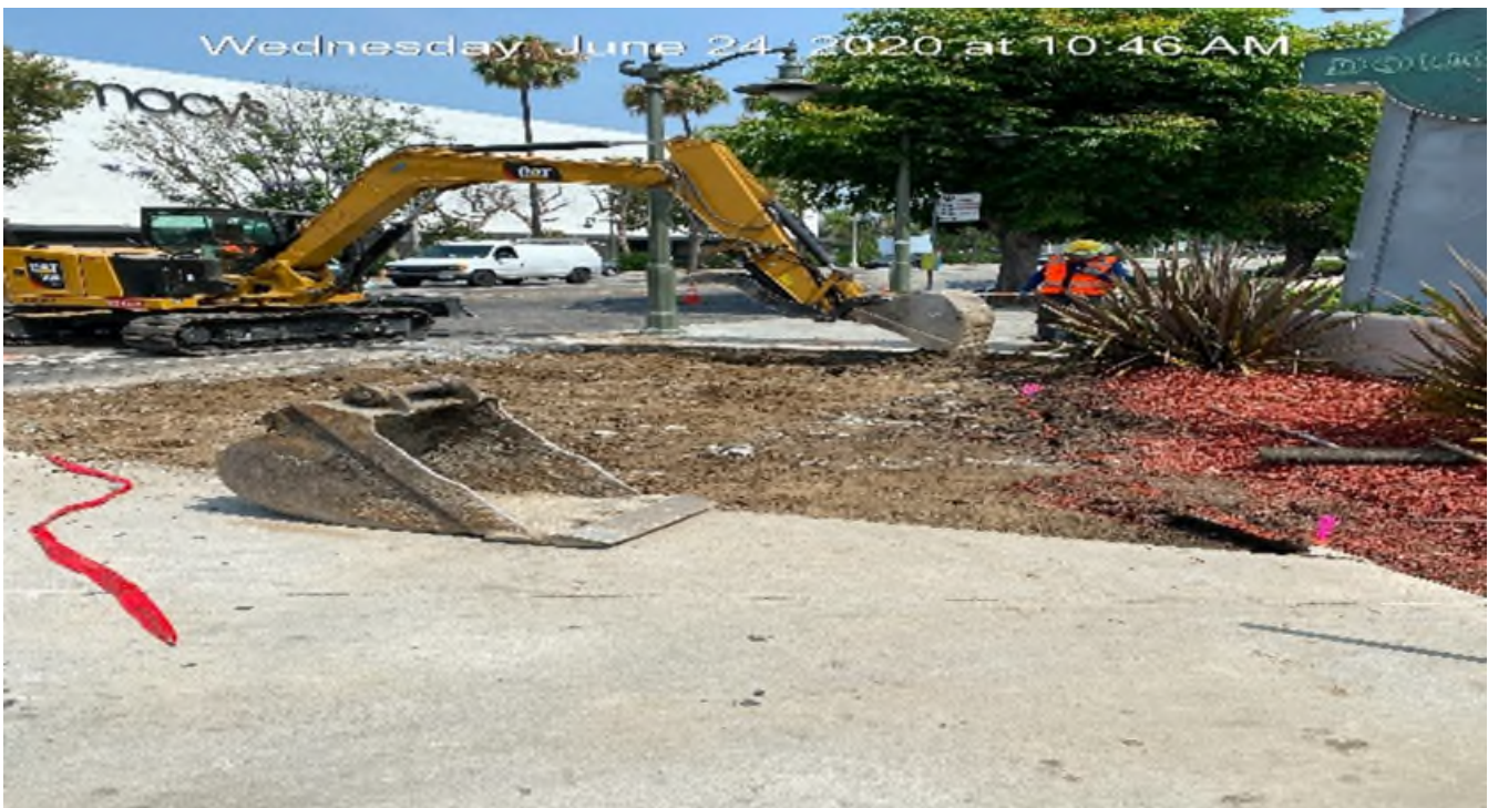
MLK STATION – Excavating/demolishing for new ADA ramp and sidewalk installation on the northeast corner of MLK Blvd and Crenshaw Blvd.
