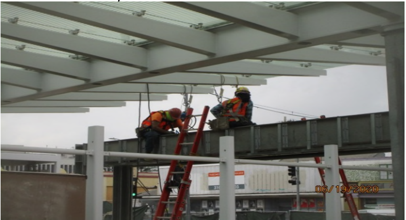
LEIMERT PARK STATION – Installing roofing deck to the main entrance canopy structure at the plaza level.
