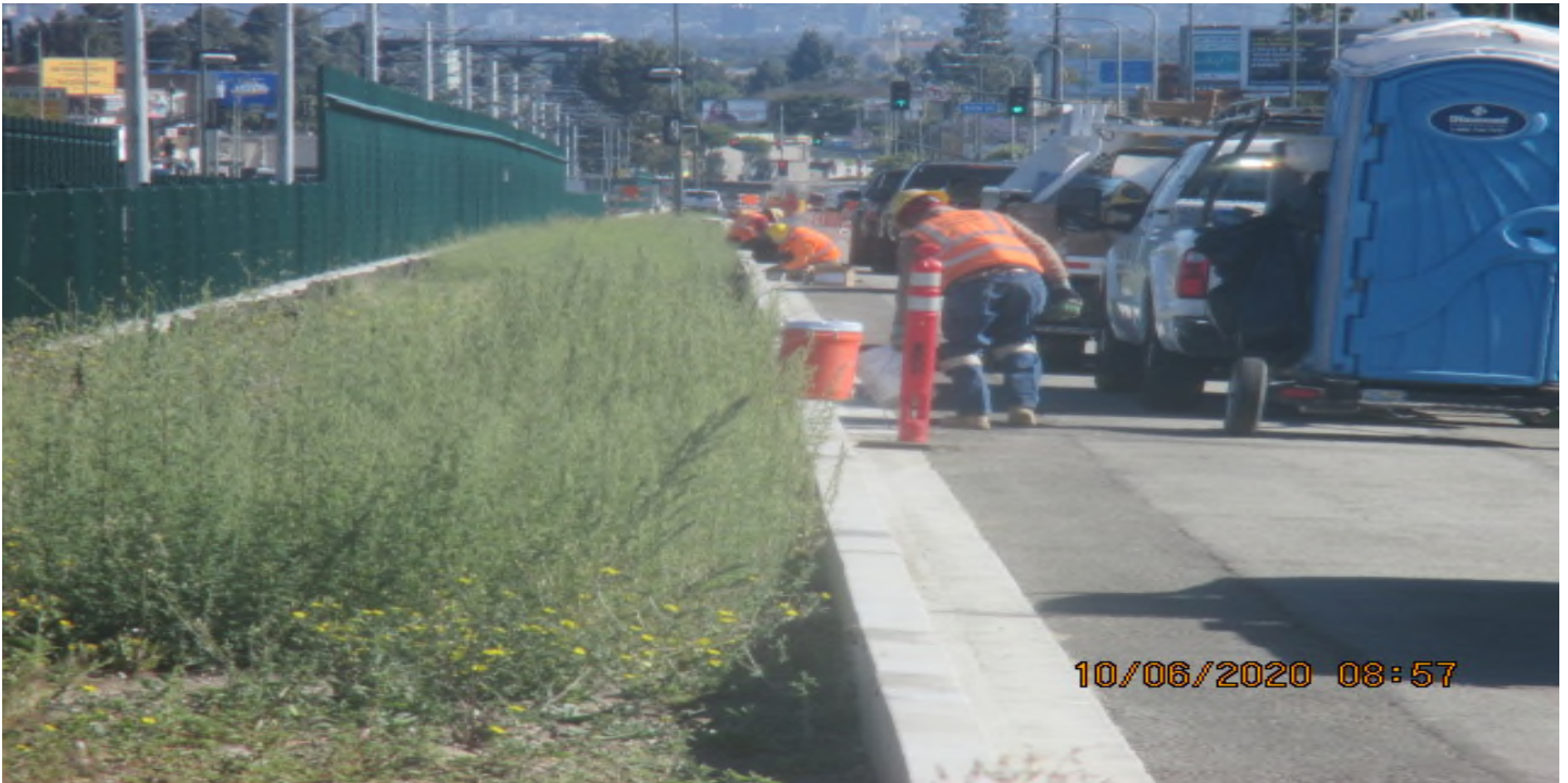
PARK MESA – Continue sack and patching center median on northbound Crenshaw Blvd between 50th St. and 52nd St. 6/10/20
