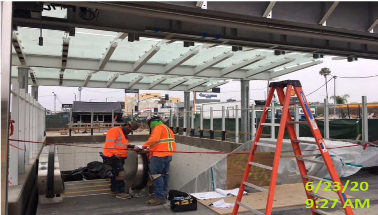
EXPO STATION – Measuring and preparing for stainless steel cladding installation for the main entrance escalators at the plaza.
