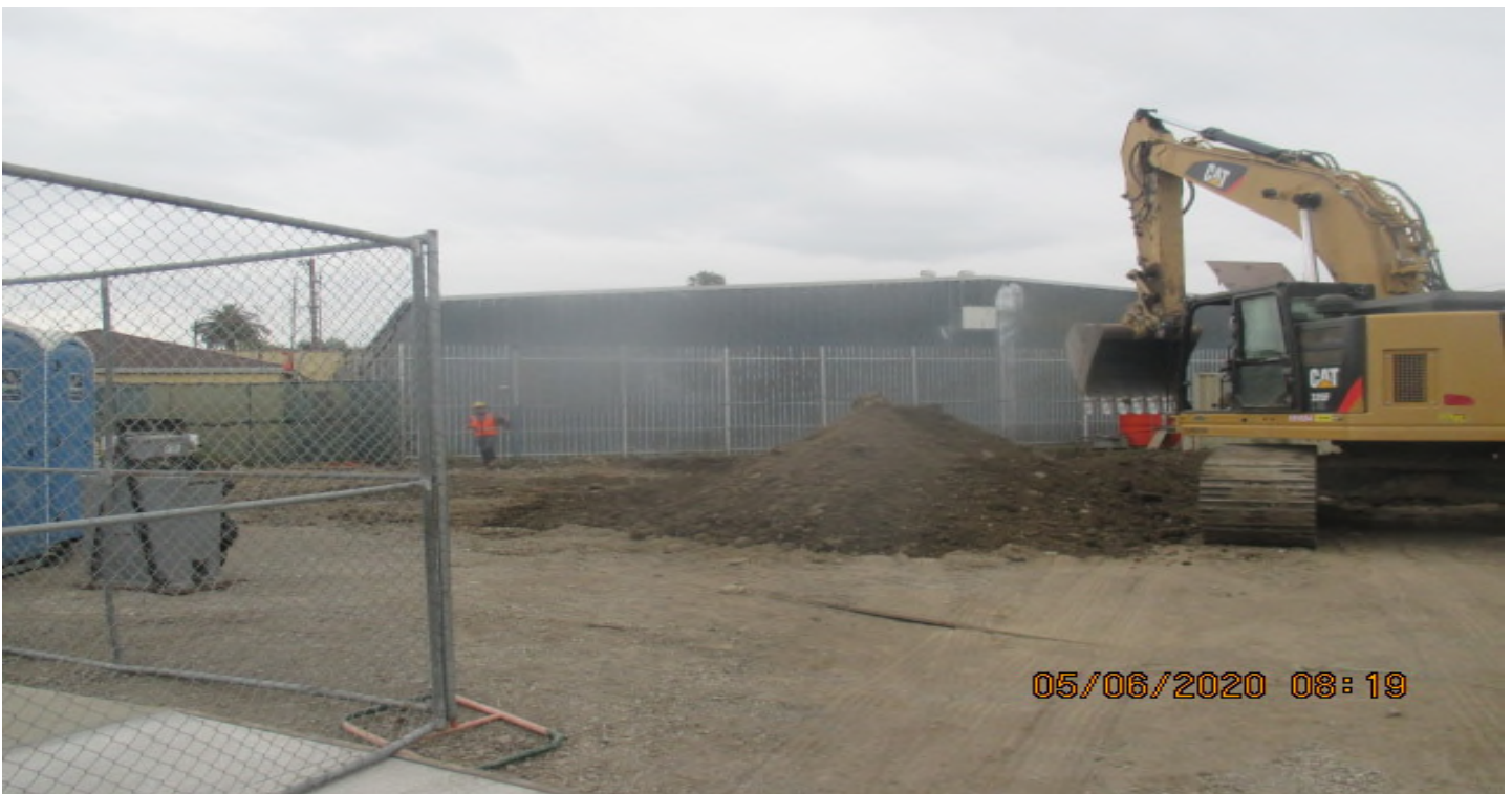
UG3 – Continue excavating/grading the north east section of Victoria Yard for upcoming pavement installation.
