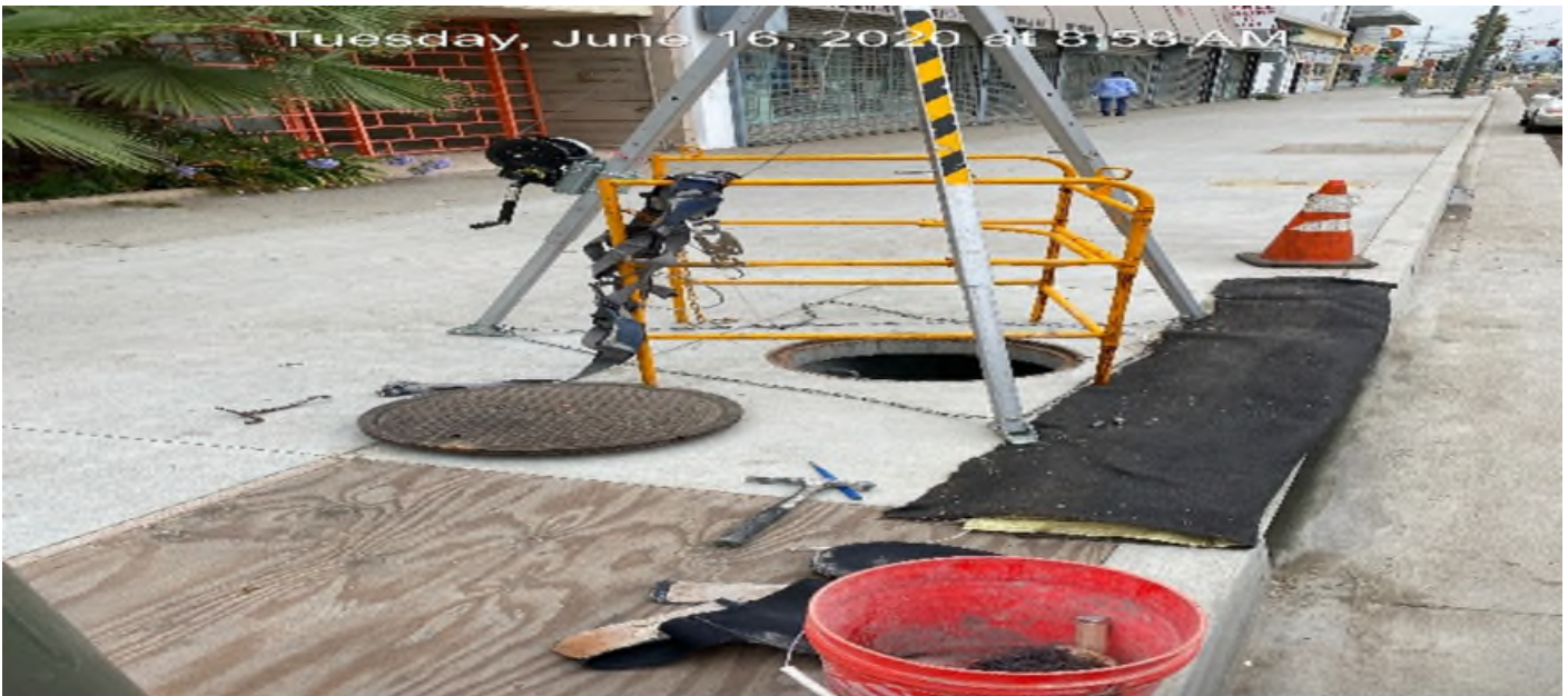
EXPO STATION – Sack and patching Catch Basin #8 on southbound Crenshaw Blvd between Rodeo Pl and Obama Blvd.
