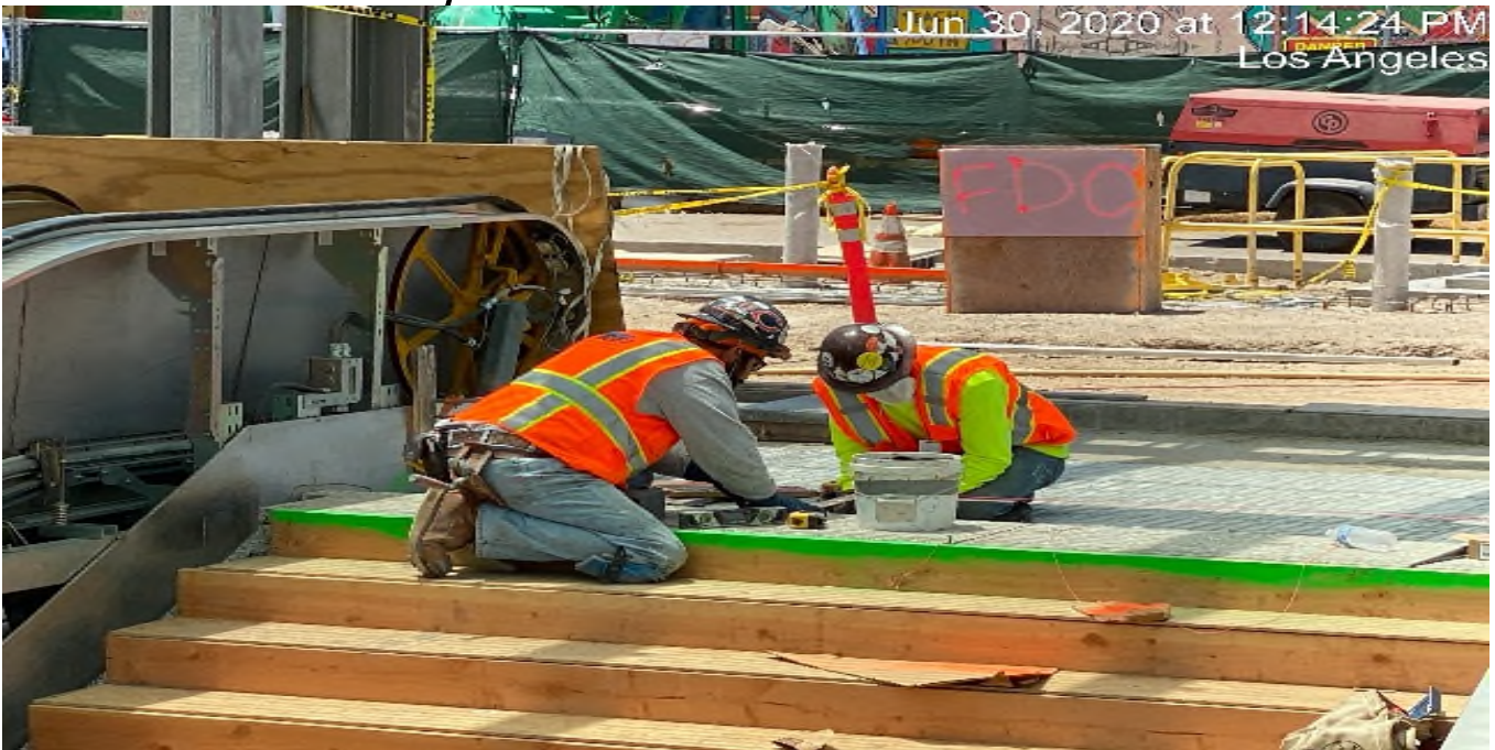
LEIMERT PARK STATION – Continue installing granite treads for the main entrance staircases at the plaza level.
