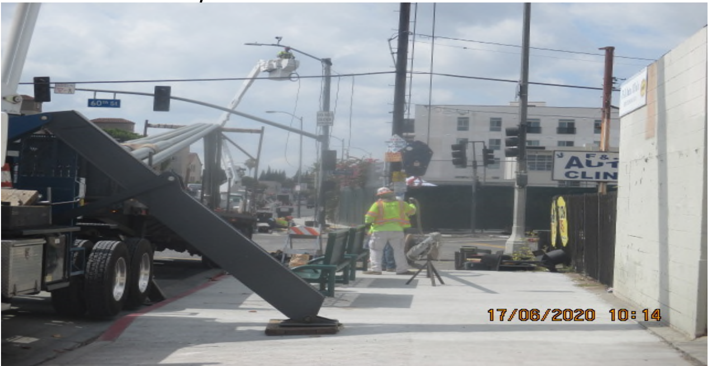
PARK MESA – Installing street light poles on both north and southwest corners of 60th St & Crenshaw Blvd. 6/17/20
