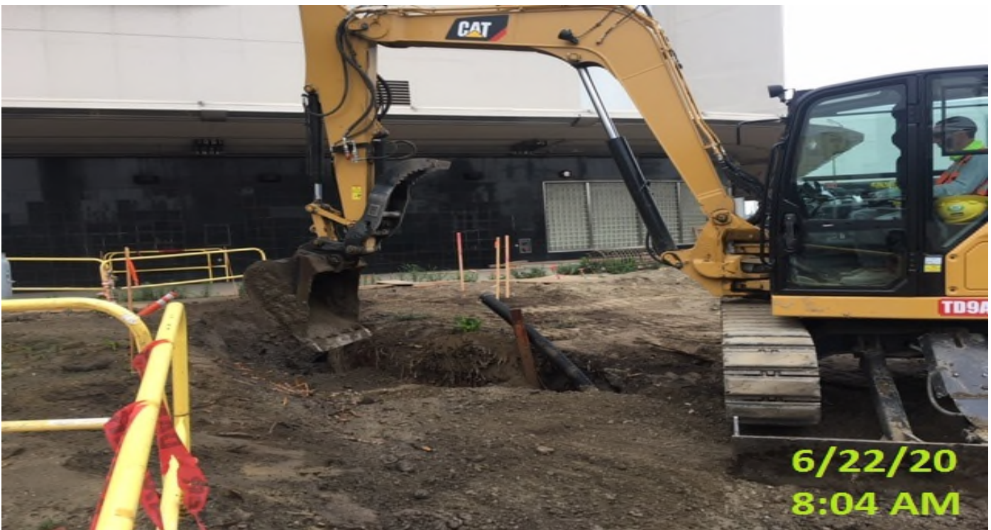
MLK STATION – Backfilling and compacting storm drain trench at the plaza level.
