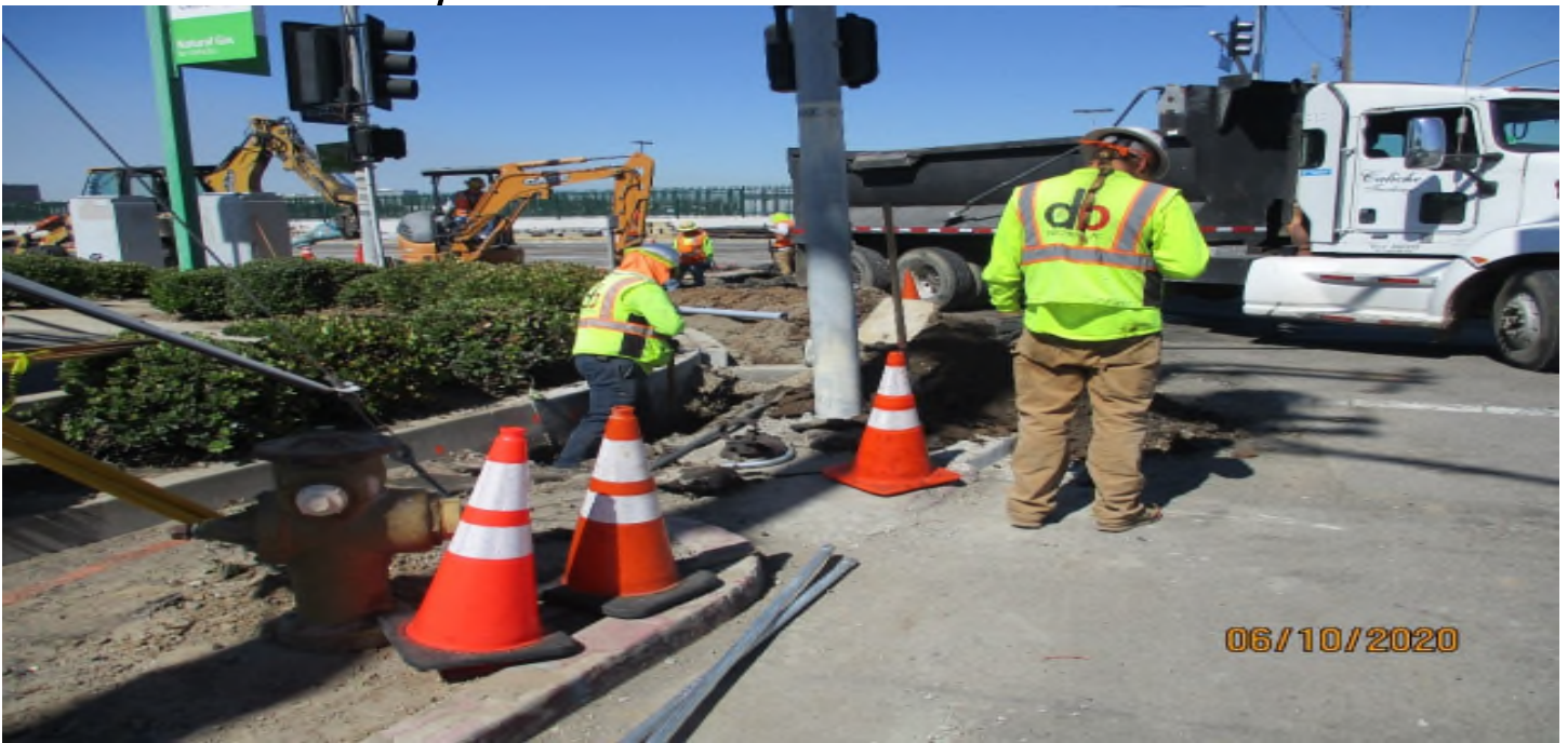
AVIATION/CENTURY- Trenching and placing conduit for streetlight pole #30 on the SE corner of the 104th & Aviation intersection. Facing SW.
