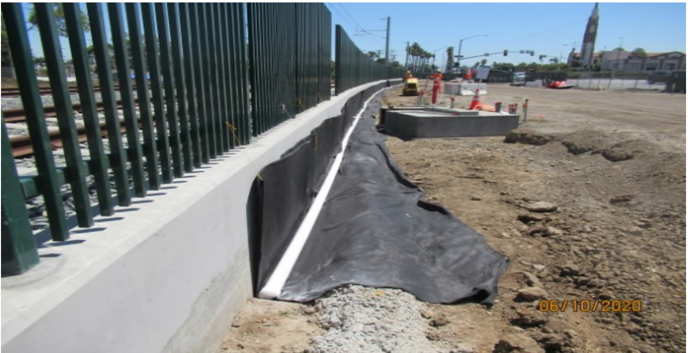
La Brea – La Brea Station WSCC preparing to Burreto rap storm drain pipe next to NB ballast retaining wall STA 156+00 (looking north)
