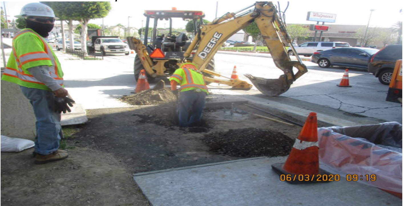
La Brea – Select Electric Excavated to place pull boxes at La Brea and Florence and under La Brea Bridge.
