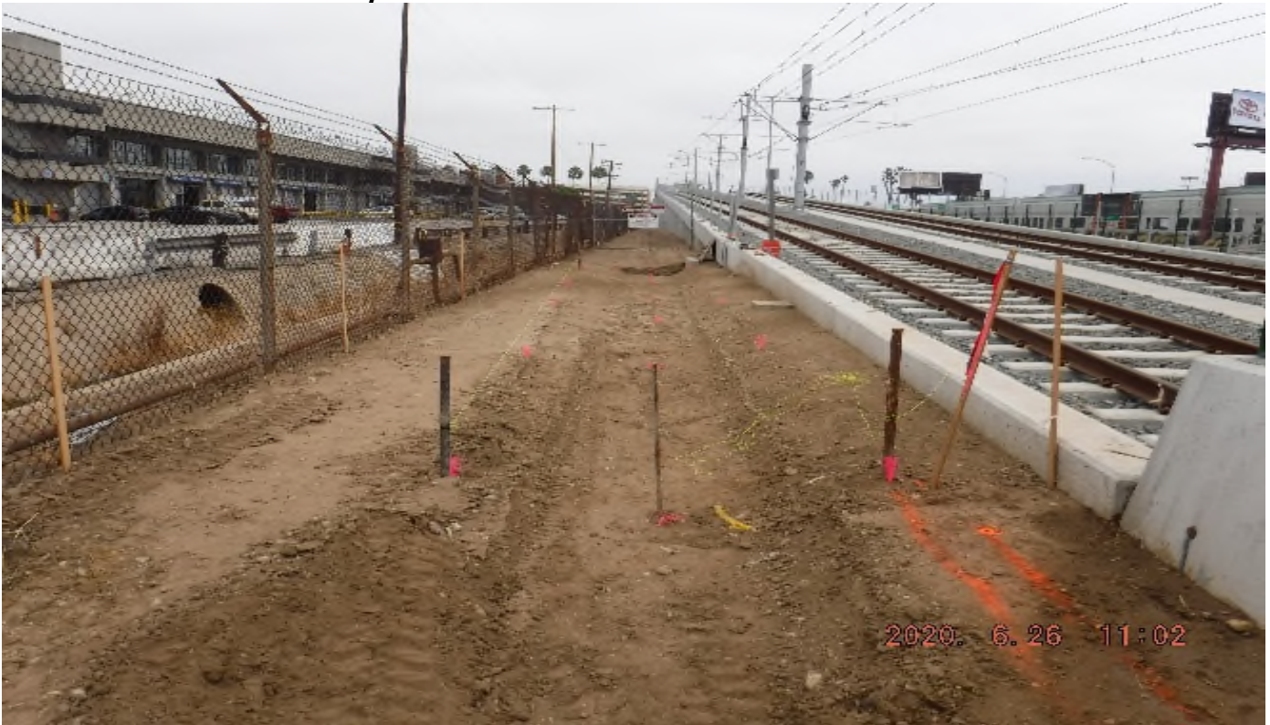
UG1- STA 59+00 looking north – grading work next UG1 “U” wall toward RW60L
