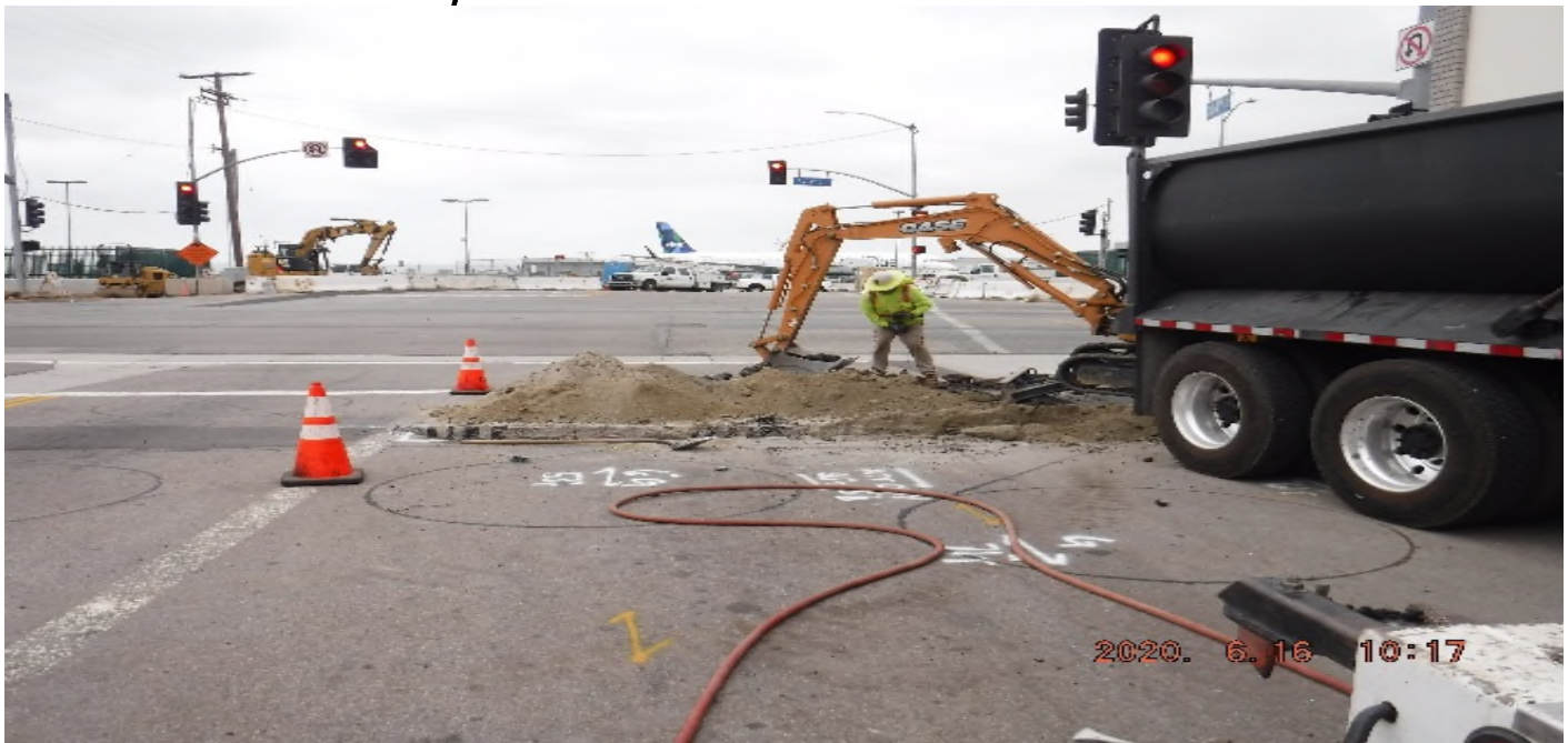
AVIATION/CENTURY- STA 55+00 looking west – trenching for traffic conduits set crossing 104th St w/Aviation Blvd.
