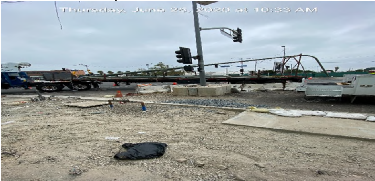
EXPO STATION – Preparing to install street light poles on the southwest corner of Obama Blvd and Crenshaw Blvd.
