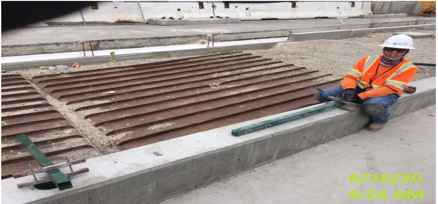
UG4 - Installing guardrail posts along both sides of the guideway curb at Sta 317+75.
