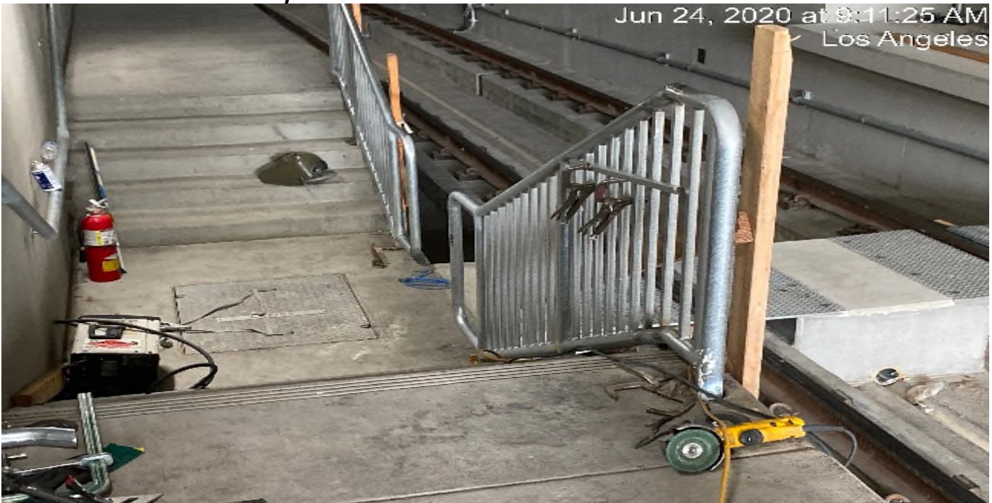
UG4 – Continue installing handrails at the south end portal and throughout the northbound tunnel.
