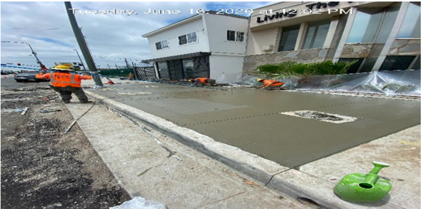
LEIMERT PARK STATION – Placing concrete for new sidewalk installation on southbound Crenshaw Blvd between 48th St and Brynhurst Ave.
