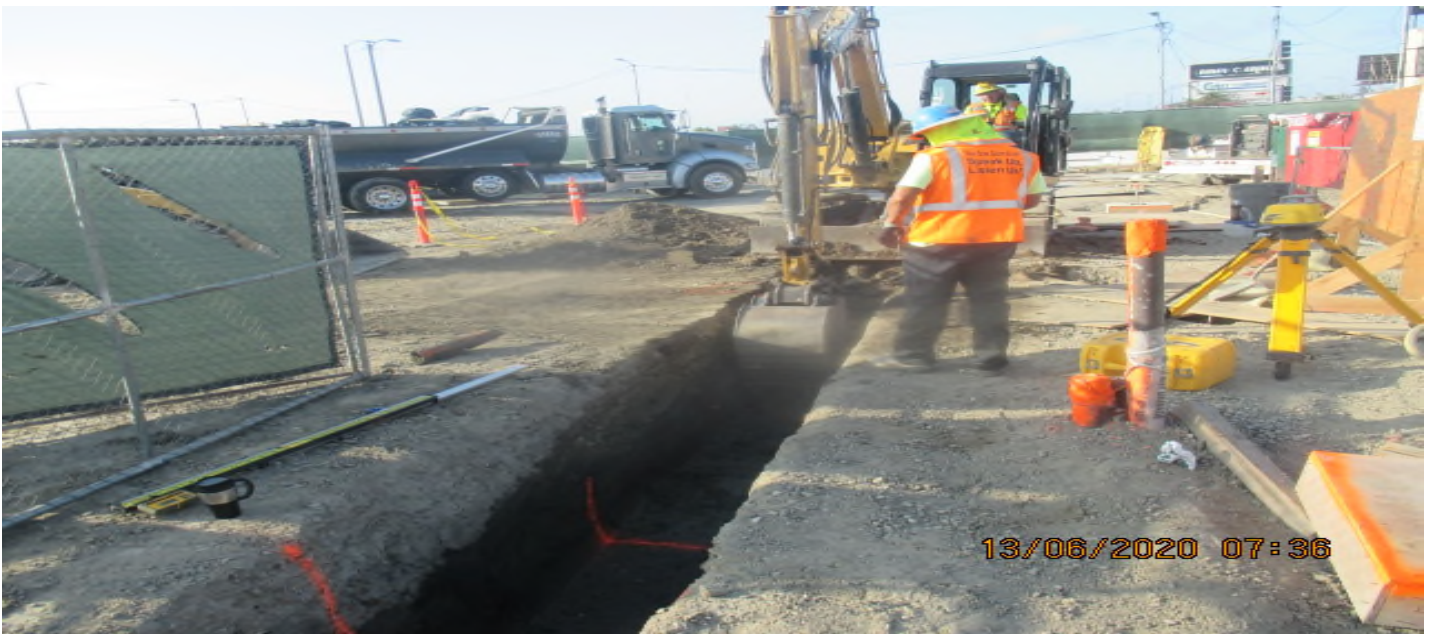
EXPO STATION – Continue excavating/trenching for underground conduit installation for landscape lighting/utilities and irrigation at the plaza level. 6/13/20
