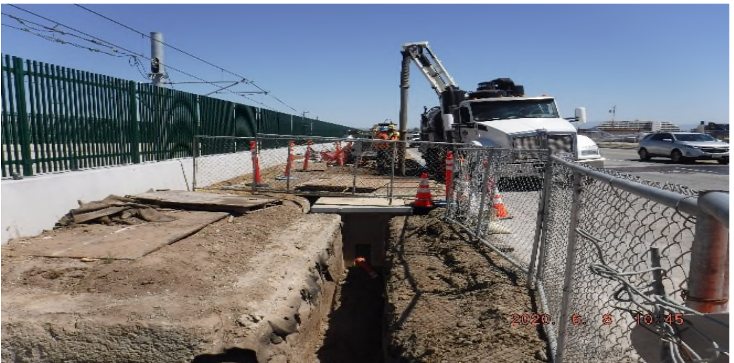
AVIATION/CENTURY- 111th Bridge area looking north (STA 33+00) – vacuum excavation subject of PCI 50505.04
