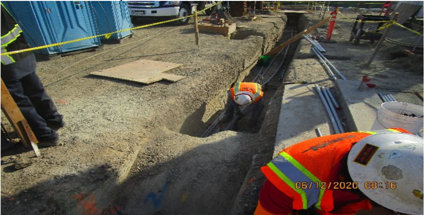
VERNON STATION- Continued rough in underground feeds (tie in) 1' schedule 40 PVC to light standard foundations stub outs.
