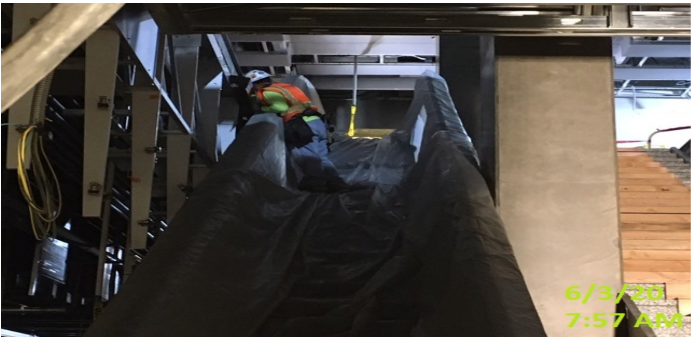
MLK – Continue installing stainless steel cladding panels on the smoke screen edges at the platform level.
