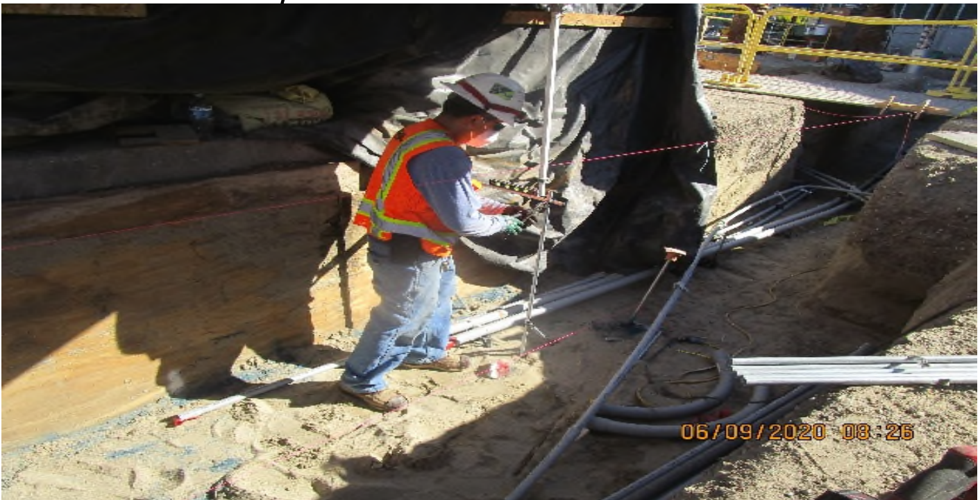
VERNON STATION- Continued rough in underground Comm power CCTV & telephone pull boxes behind elevators 1 & 2.
