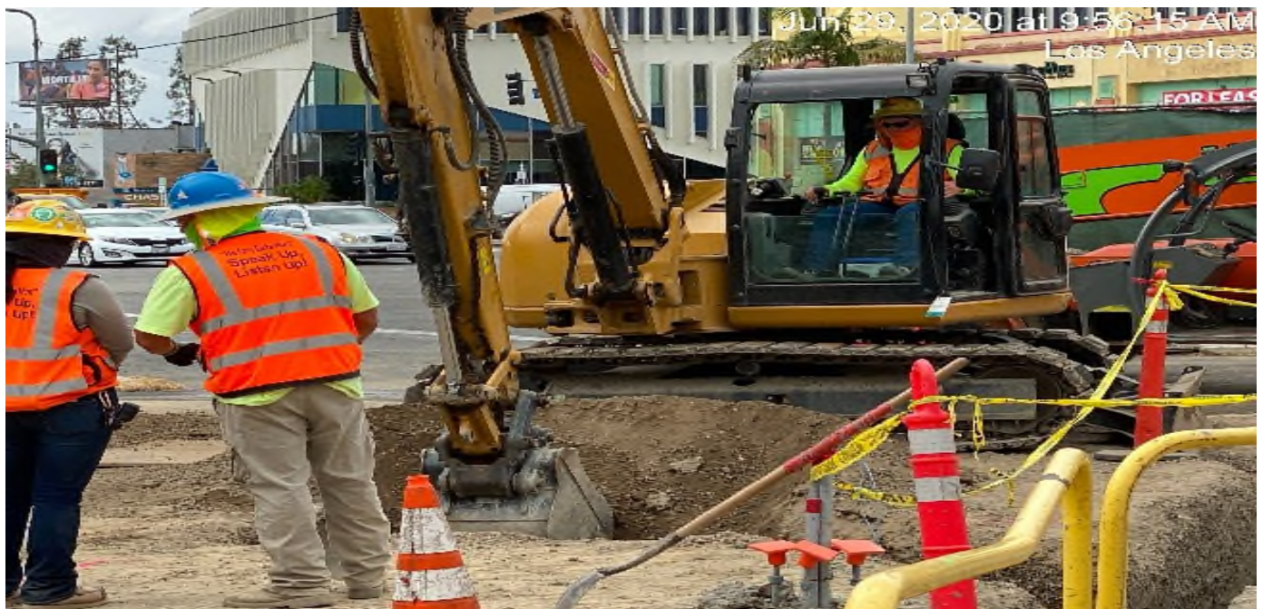
LEIMERT PARK STATION – Excavating for grand pylon foundation at the southeast corner of the plaza level.
