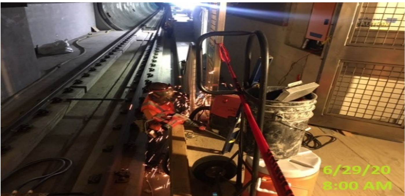
MLK STATION – Continue installing guardrails for both south and northbound tunnels at the south end invert level.
