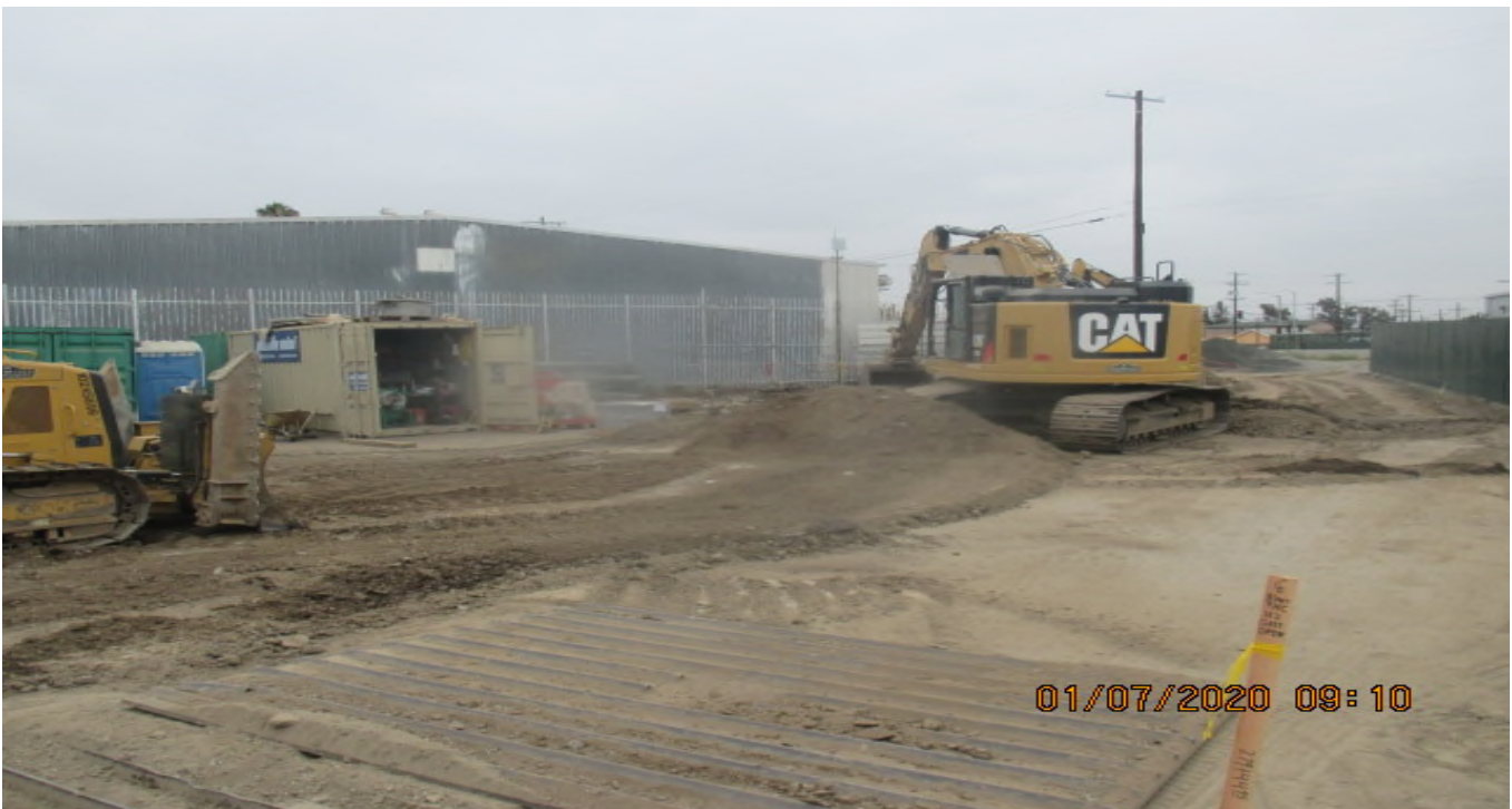
UG3 – Continue excavating/grading the remaining area of Victoria Yard and preparing for granite base rock placement. 7/1/20
