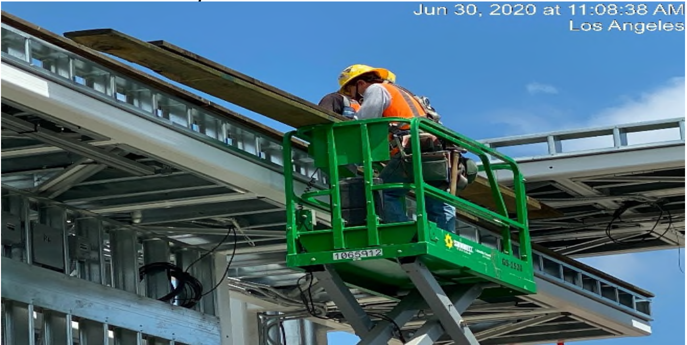
HYDE PARK STATION – Continue forming roof for the north canopy structure at the platform.
