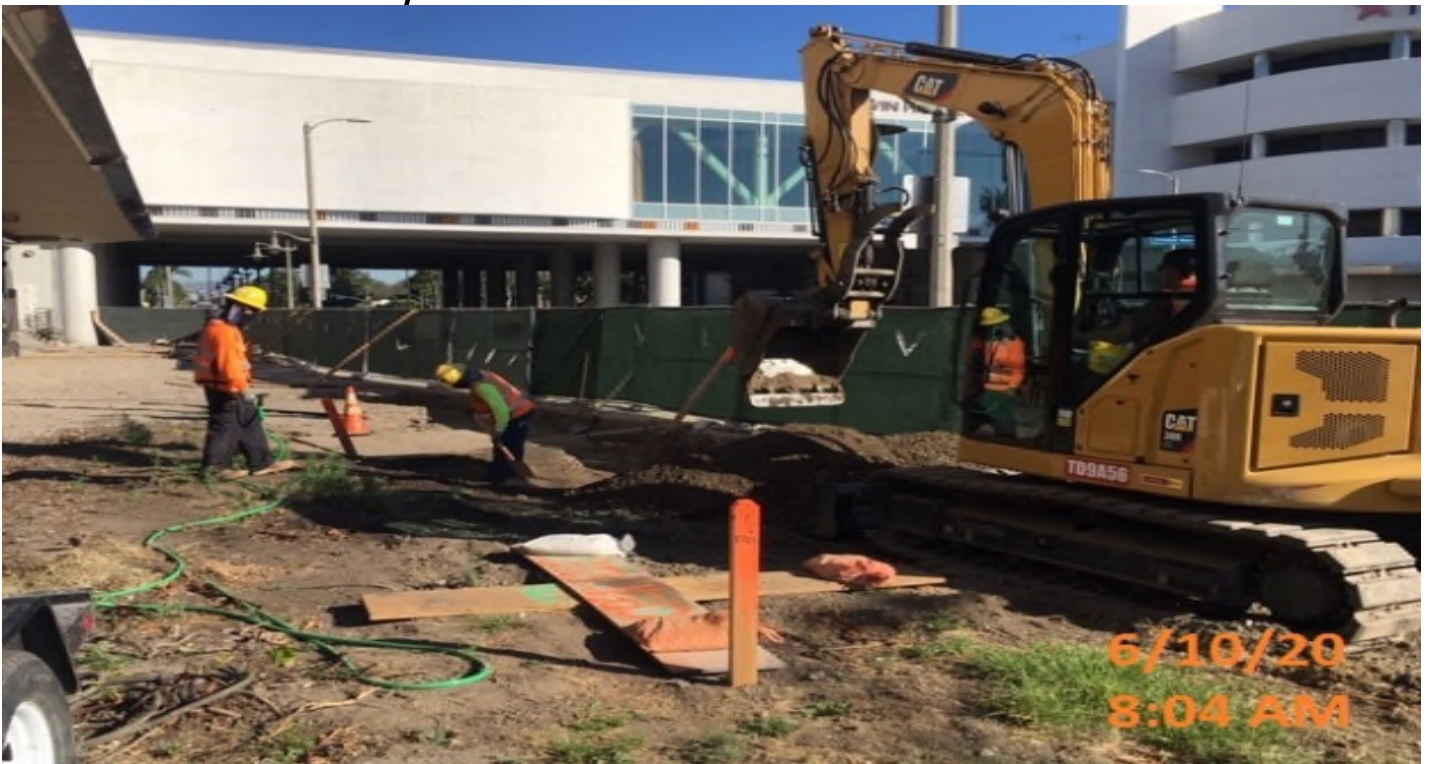
MLK - Excavating for upcoming paver and sidewalk installation at the north end of the plaza level.
