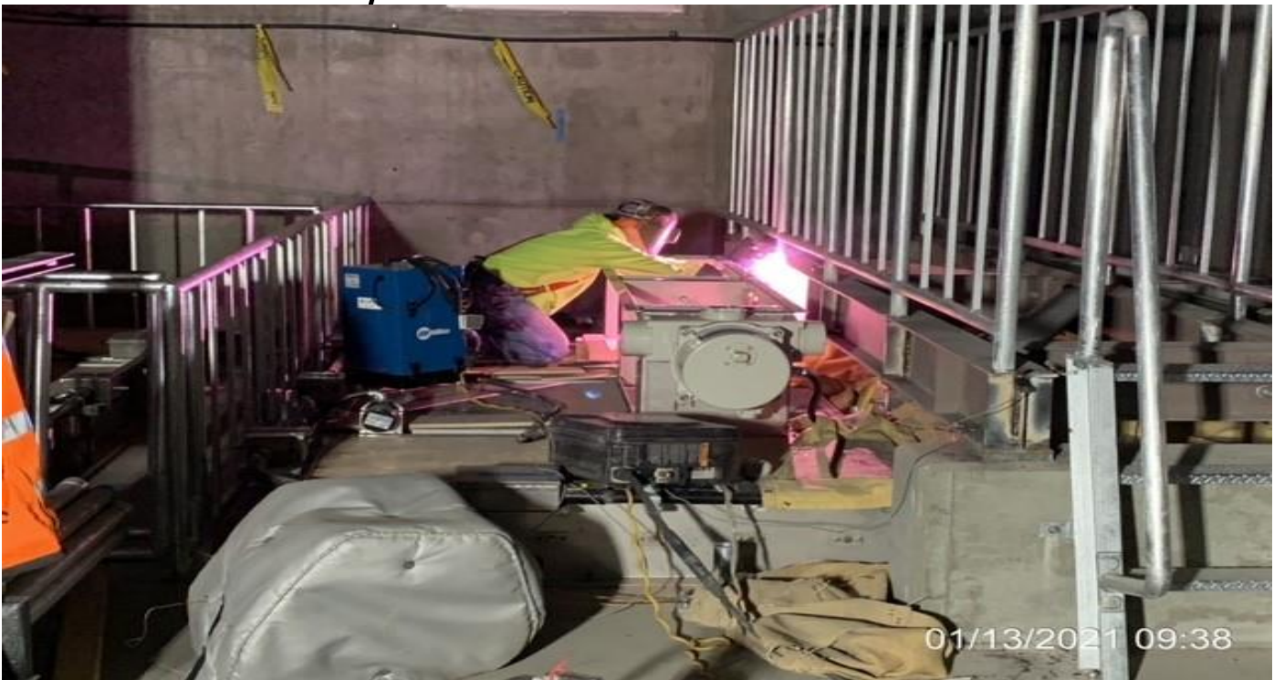
MLK STATION – Installing stiffener plates for the guardrails inside the Emergency Ventilation Shaft/OTE Plenum South C-101.
