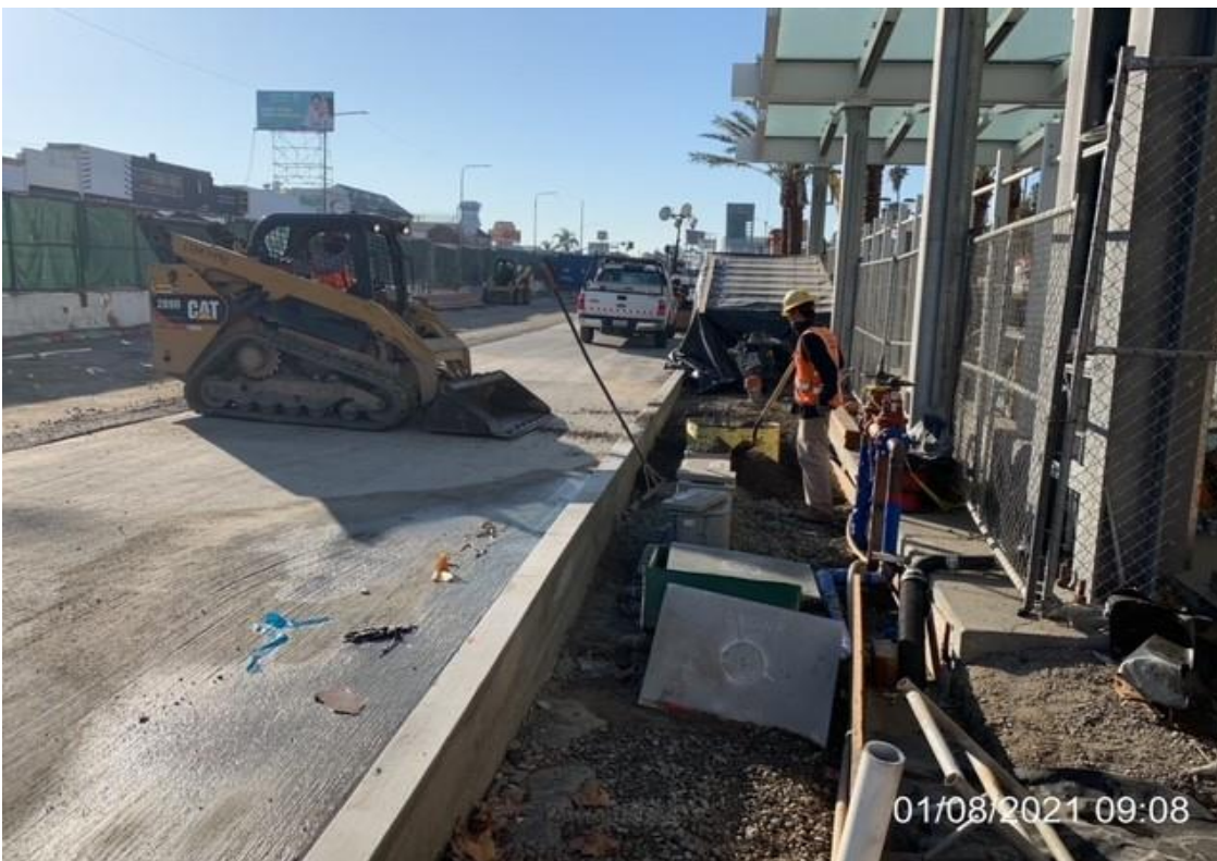
MLK STATION – WSCC crew backfilling with base along curb at east side of station.
