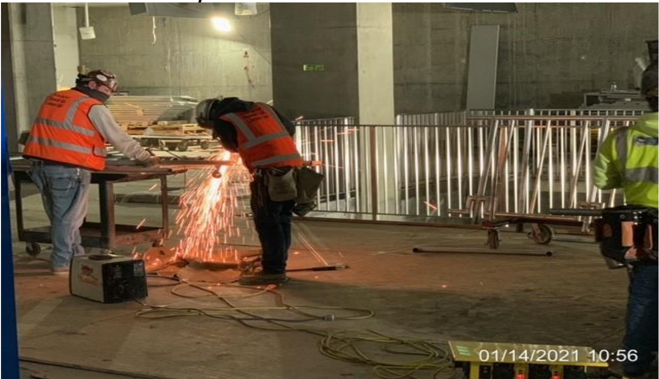
EXPO STATION – Fabricating guardrails for installation inside the Emergency Ventilation Shaft/OTE Plenum North C-126.
