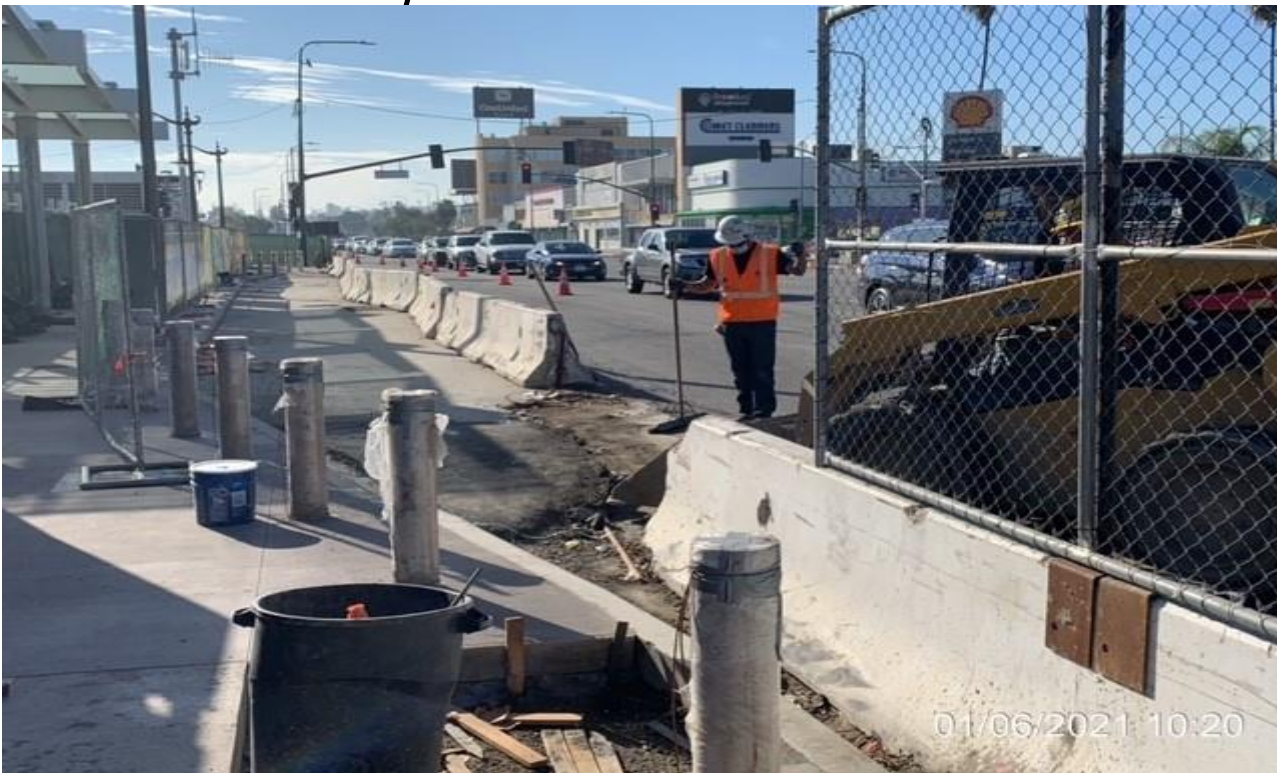
EXPO STATION – Removing K-rail in preparation for new sidewalk installation along the west of the plaza.
