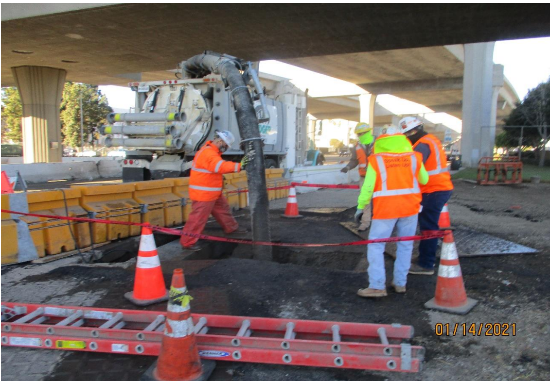
AVIATION/CENTURY- Vacuum truck exposing the Tosco line for hot tapping on Imperial at Aviation.
