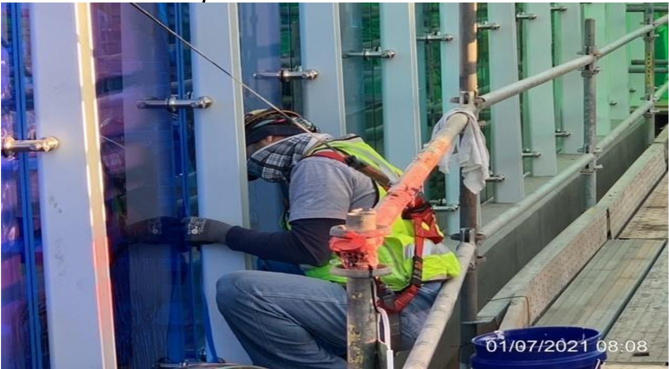
LEIMERT PARK STATION – Caulking and sealing between art glass panels around the main entrance canopy at the plaza.
