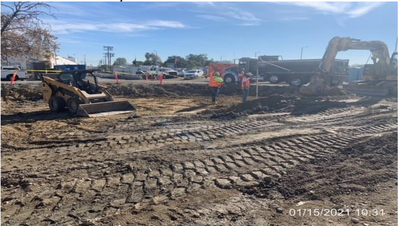
EXPO STATION – Continue rough grading and removing existing concrete on the east side of the Park & Ride lot area.
