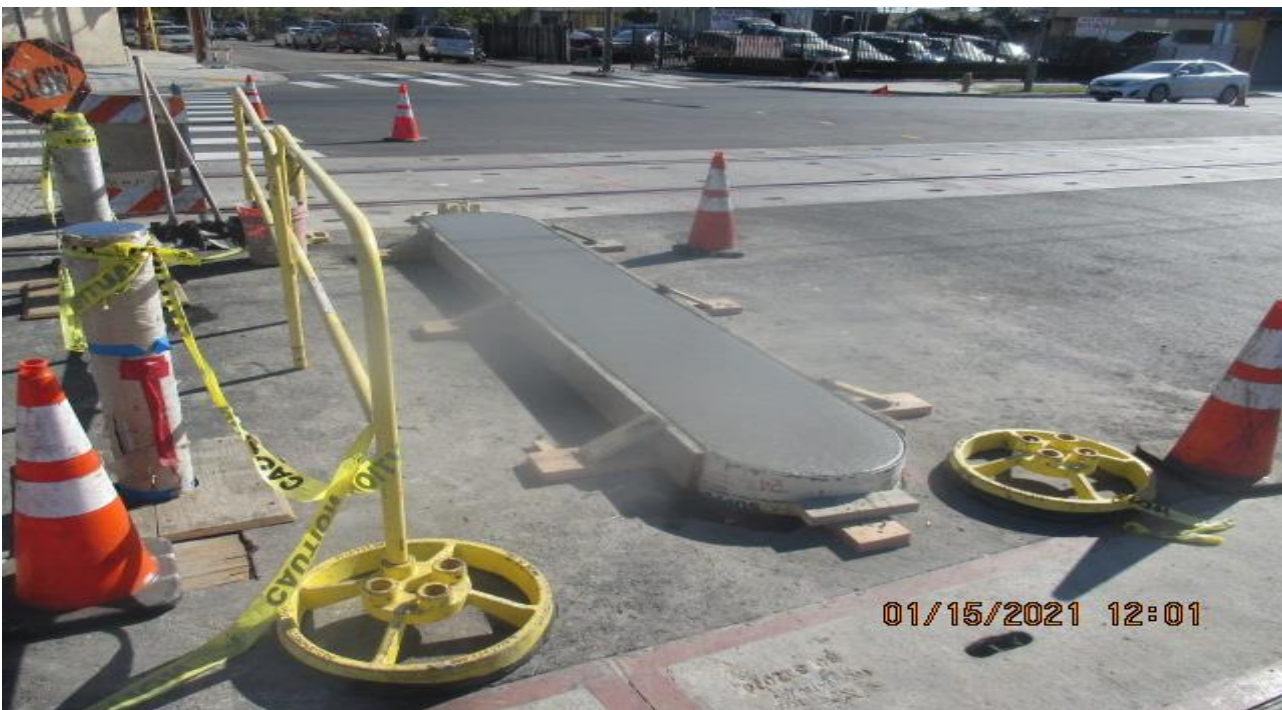
PARK MESA – Placed concrete for safety curb footings on both the north and south end crosswalks at Slauson Ave and 59th St.
