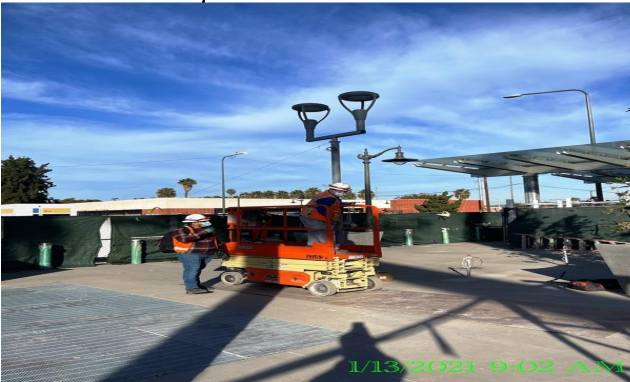
EXPO STATION – Installing CCTV camera supports to all the pedestrian light poles at the plaza.
