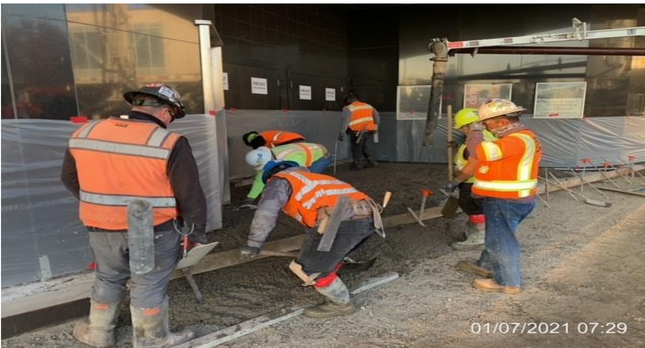
MLK STATION – Placing concrete along the north side curb of the Mall and at the two entrances
