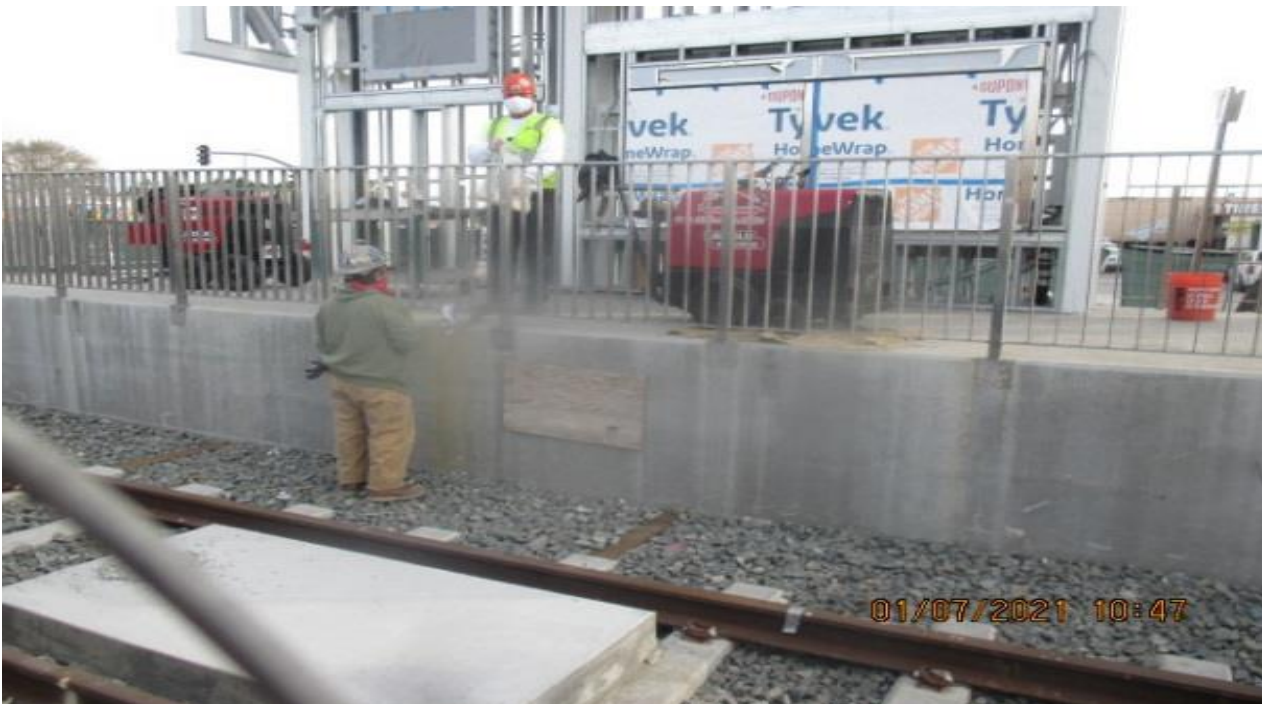
PARK MESA – Grinding and polishing handrail and guardrail finishes at the north entrance walkway ramp.
