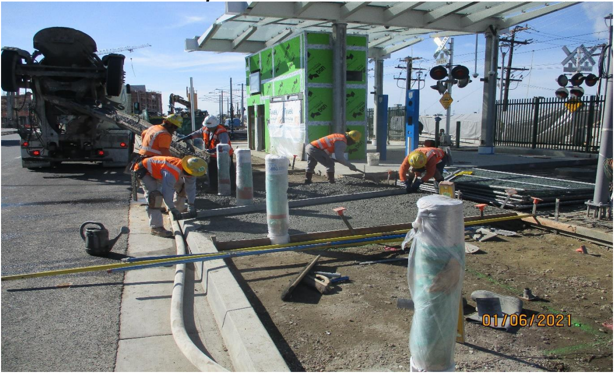
La Brea Station - Placing sidewalk concrete at the La Brea Station east TVM.
