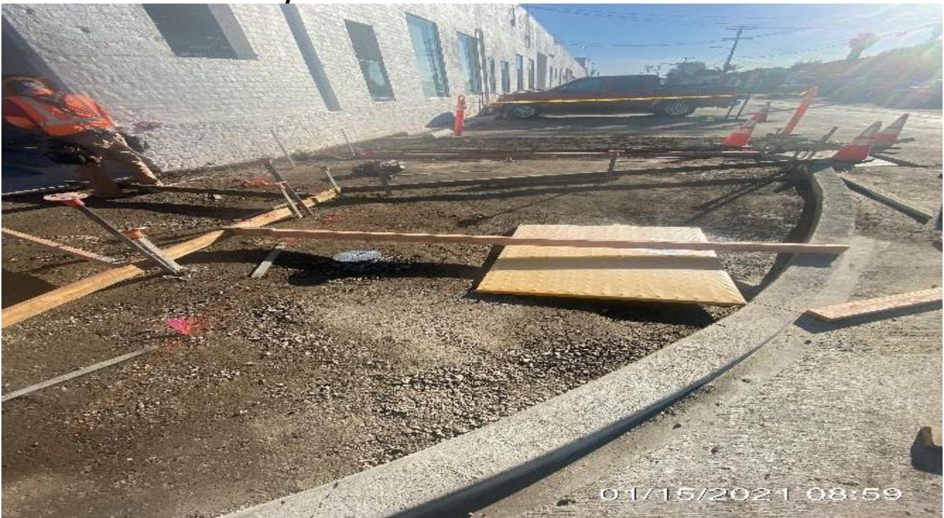
EXPO STATION – Building formwork for new ADA ramp on the northeast side of the Bronson Cul-de-sac.
