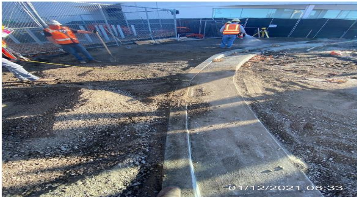
EXPO STATION– Continue excavating to final grade at the northbound sidewalk along the Bronson Cul-de-sac.
