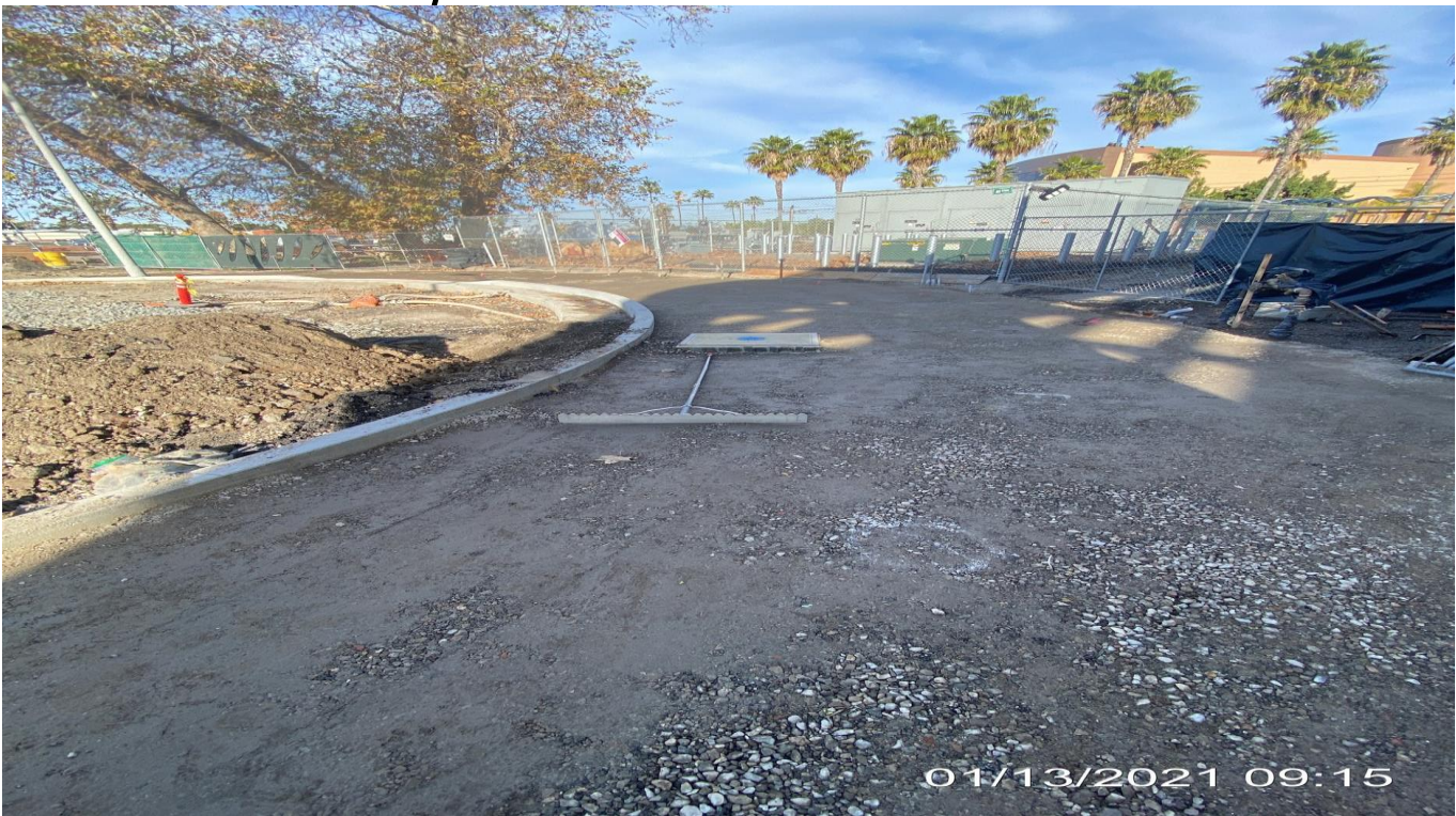
EXPO STATION SITE – Continue excavating to final grade at the northbound sidewalk along the Bronson Cul-de-sac.
