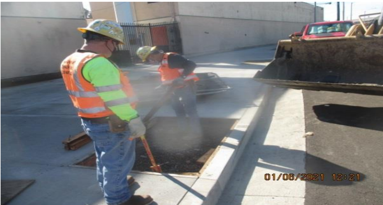
UG3 – Placing top soil to tree wells along the sidewalk on eastbound “New Road” and Crenshaw Blvd.
