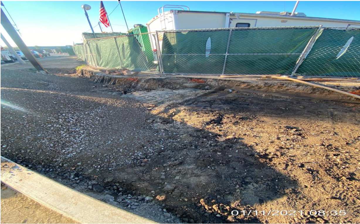
EXPO STATION– Continue excavating to final grade at the southbound sidewalk along the Bronson Cul-de-sac.
