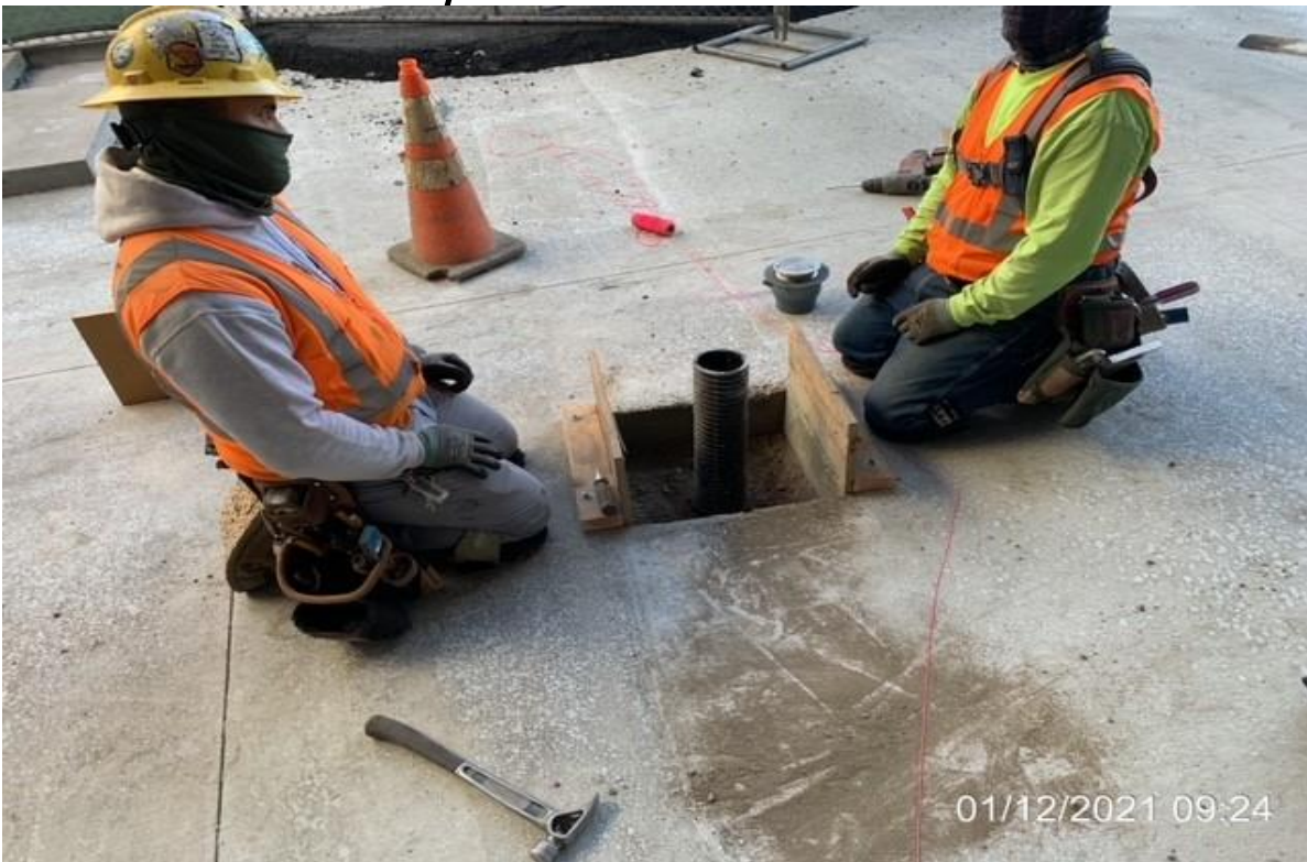
MLK STATION – WSCC carpenters installing clean outs at north end of station.
