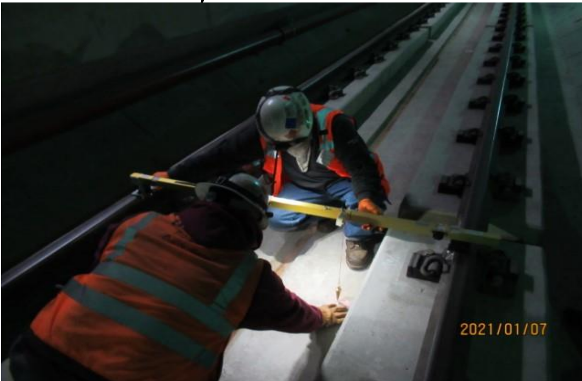
UG4 – HCC in UG4 on SB-36 curve verifying correct alignment using survey scribe nail & plum bob (looking south) Rework
