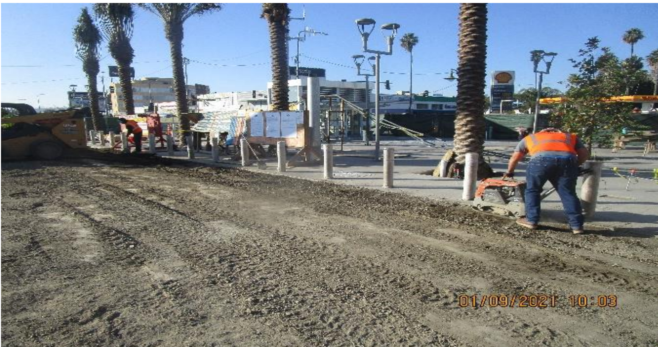
EXPO STATION – Graded/backfilled and compacted the east side of the plaza for drainage swale installation.
