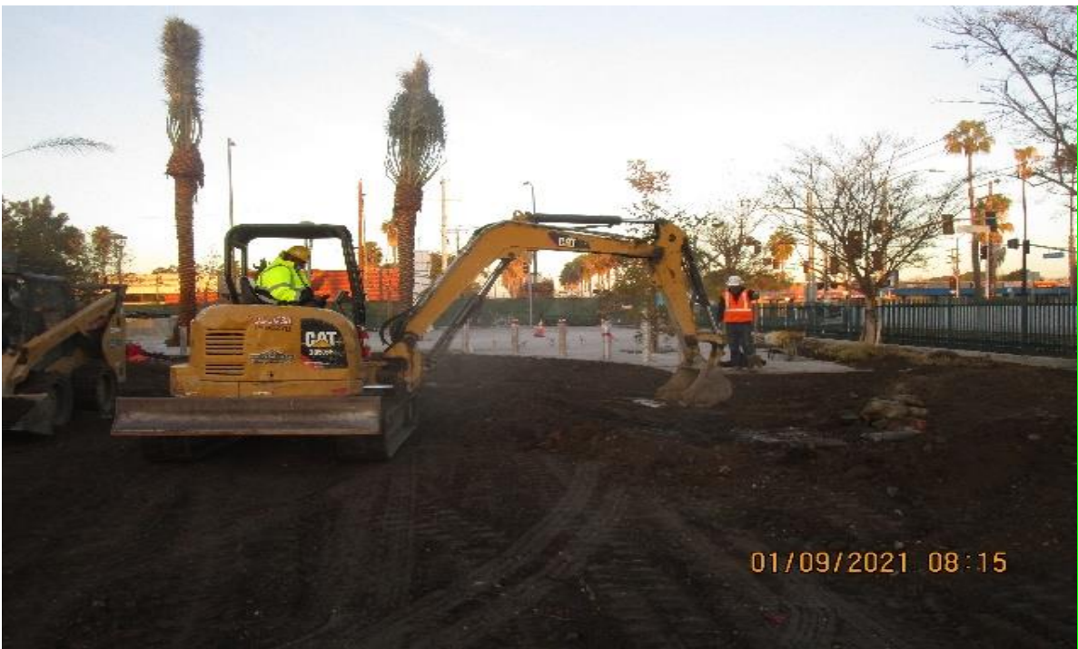
EXPO STATION – begin rough grading slop to drain at beginning of treatment swale #3 east of bollards.
