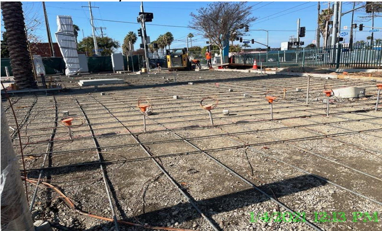
EXPO STATION – Continue ground grid installation at the north side of the plaza.
