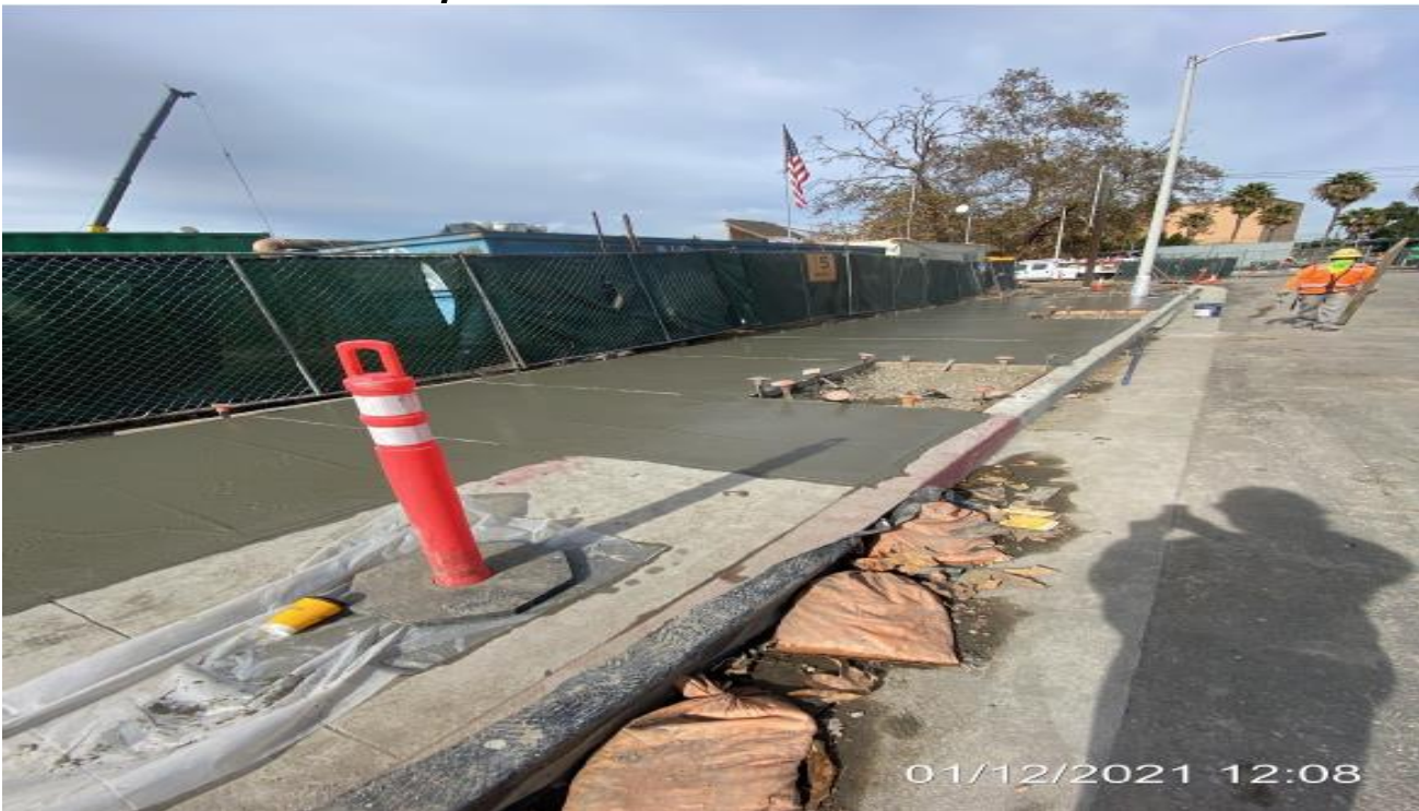
EXPO STATION – Placing concrete for new southbound sidewalk along the Bronson Cul-de-sac.
