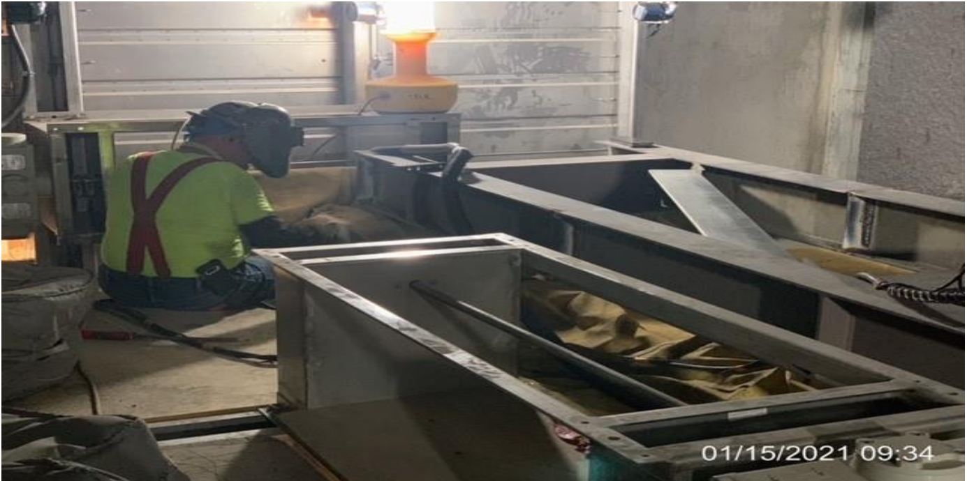
MLK STATION – Installing stiffener plates for the guardrails inside the Emergency Ventilation Shaft/OTE Plenum North C-143.
