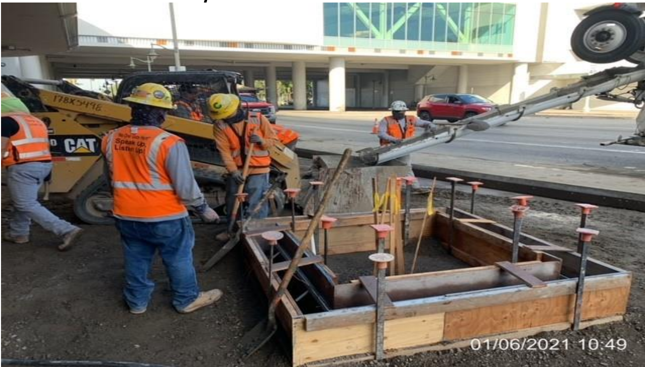
MLK STATION – Placing concrete for the tree base curbs at the far northwest area of the plaza.
