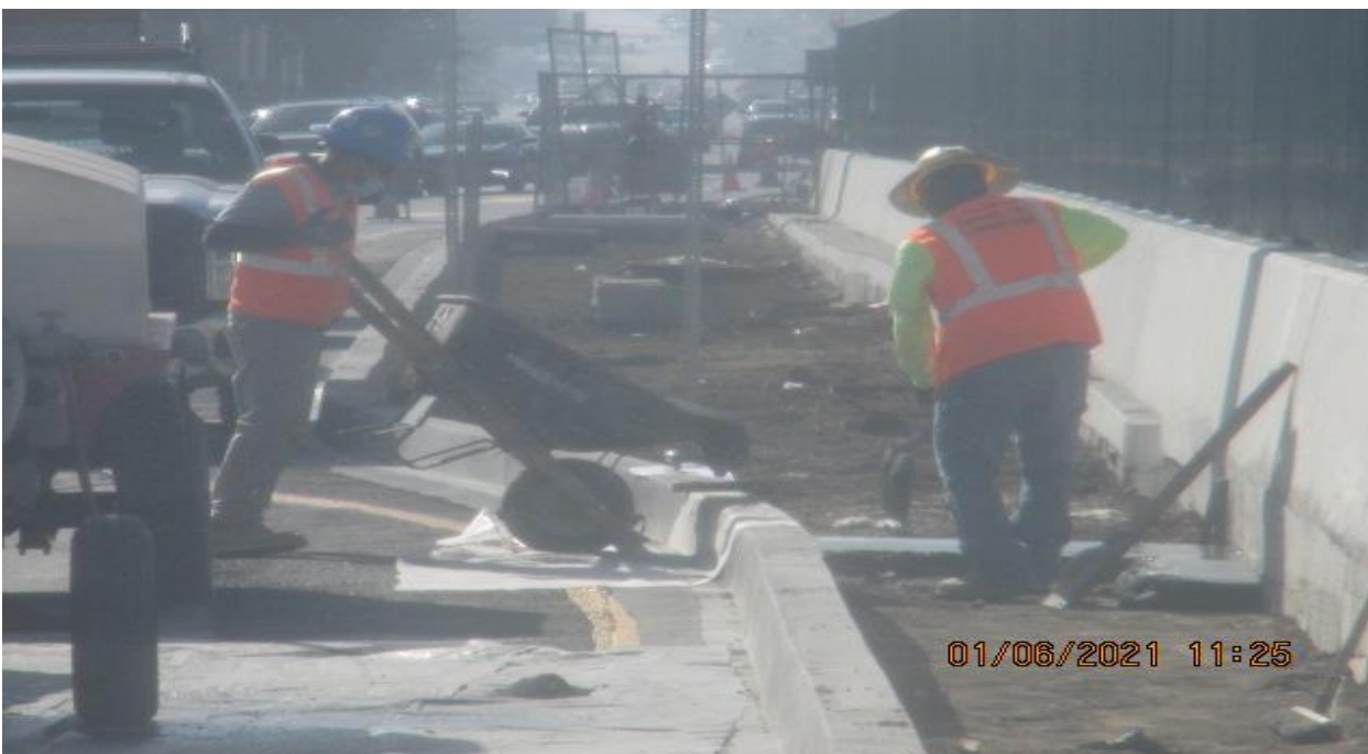
PARK MESA – Continue mixing and placing mortar base for cobble installation on the northbound median curb on Crenshaw Blvd from 59th Pl to 59th St.
