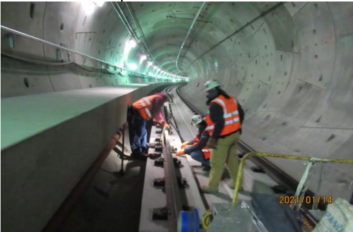
UG4 – HCC in UG4 NB track adjusting super elevations on NB-33 394+25 (looking north) Rework.
