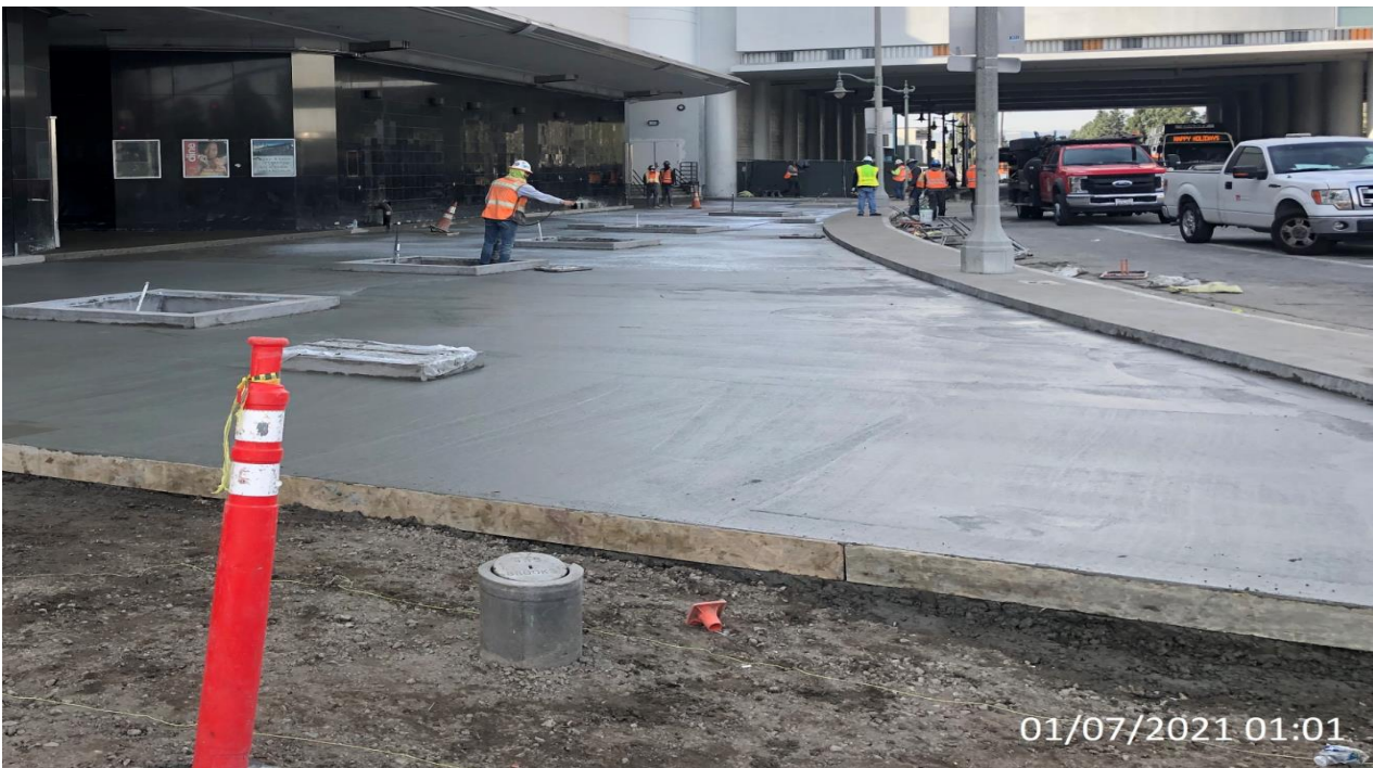
MLK STATION – Spraying curing compound to the entire concrete slab on the northwest section area.
