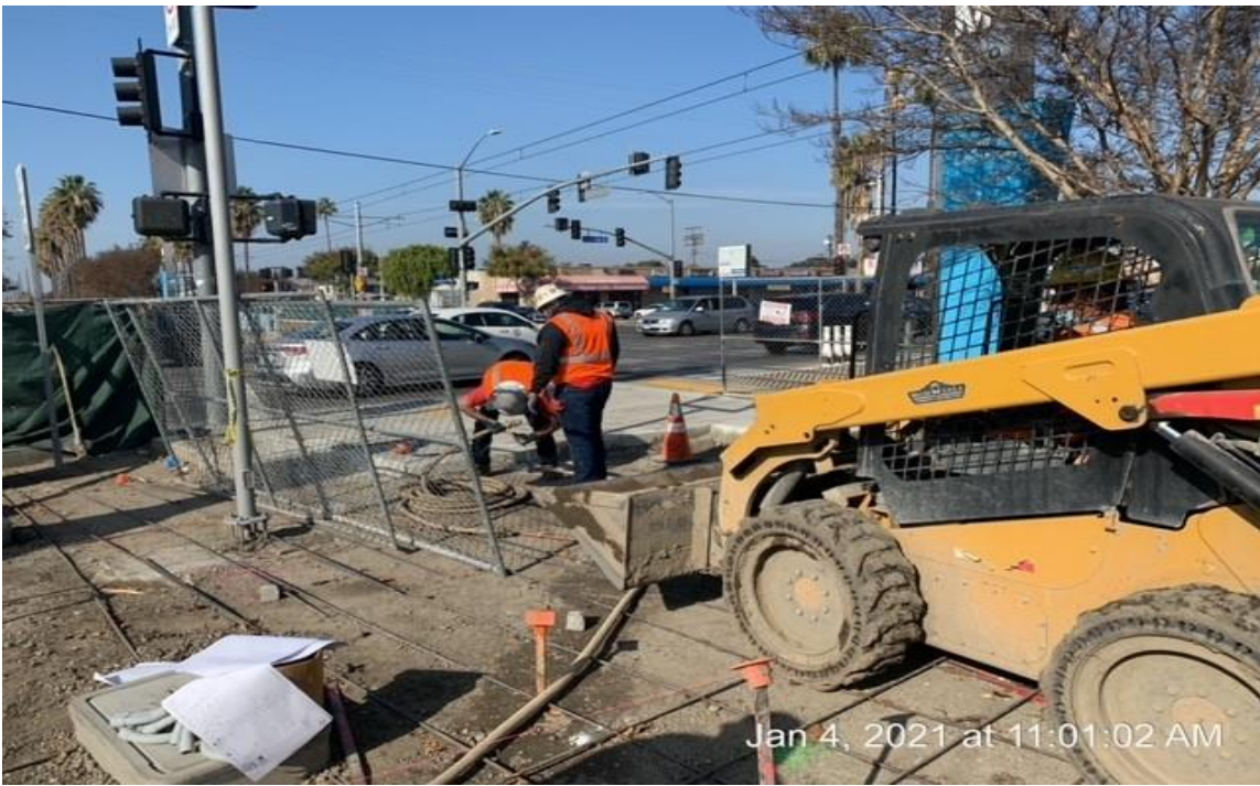
EXPO STATION - Removed existing concrete sidewalk at the northwest corner of the plaza.
