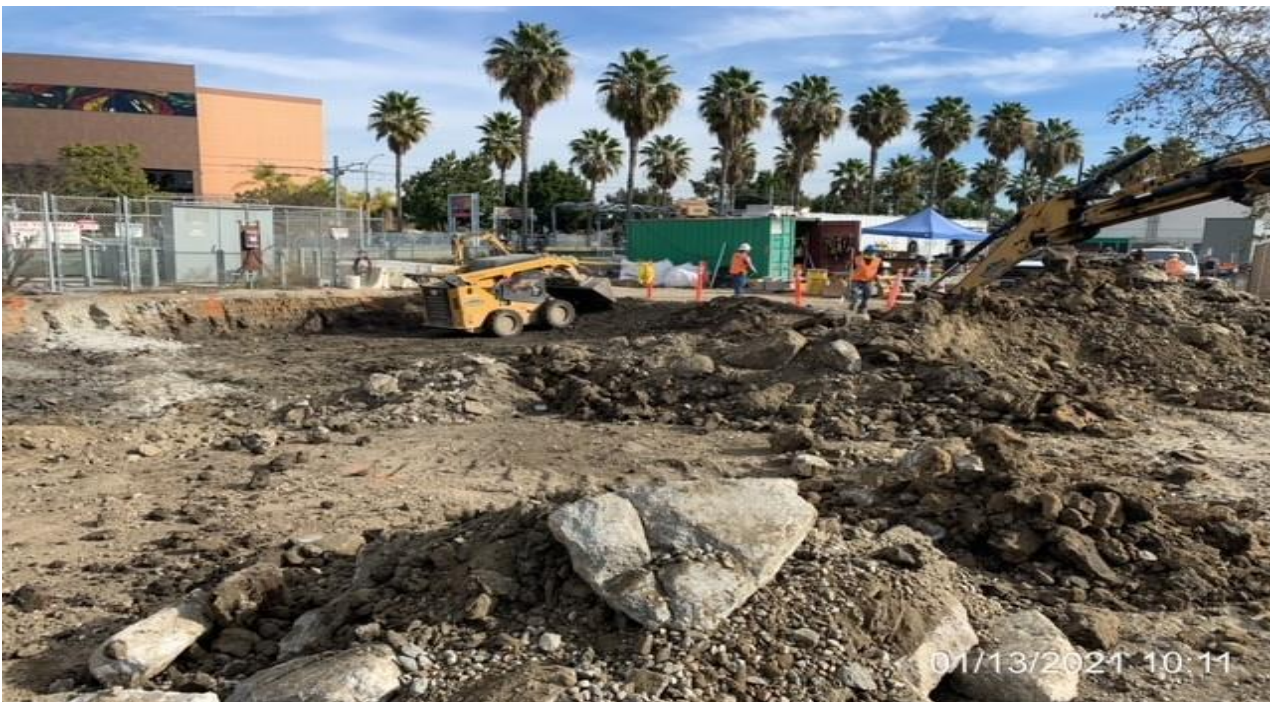
EXPO STATION SITE– Continue rough grading the northwest side of the Park & Ride lot area.
