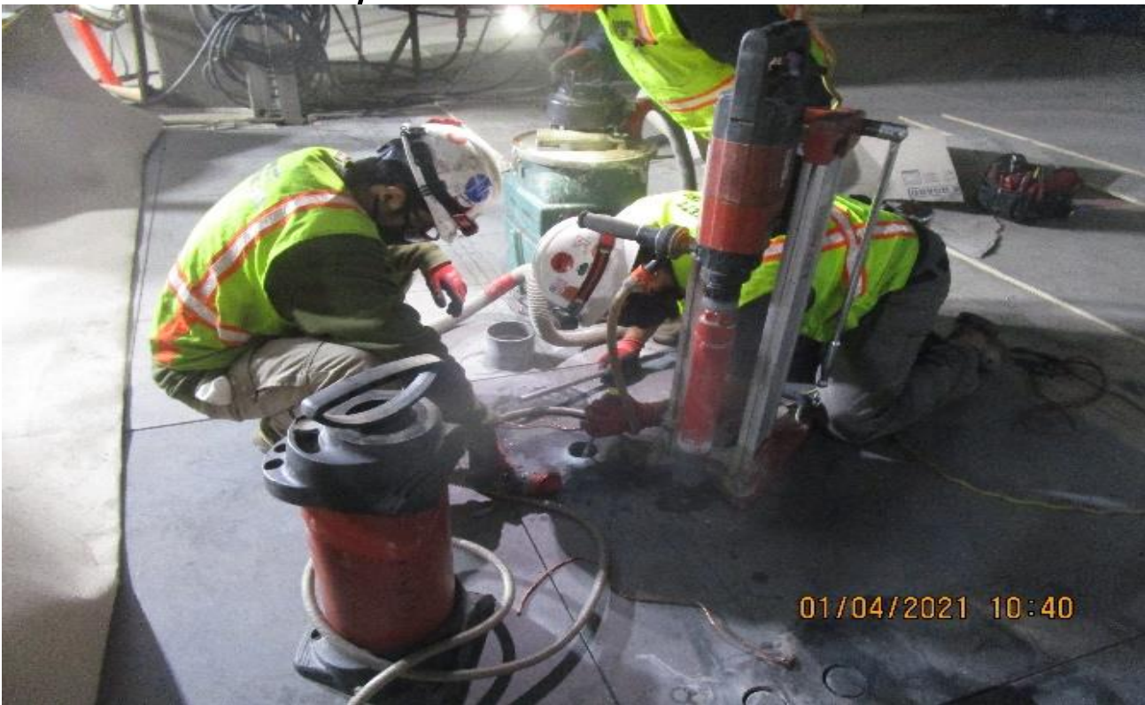
MLK STATION – Performing layout and coring through the walker ducts in preparation for the turnstile fare gate system installation at the Paid & Free Area.
