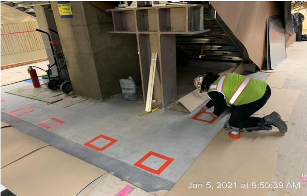
MLK STATION – Penhall prep and layout prior to coring for posts beneath stairs and escalators.
