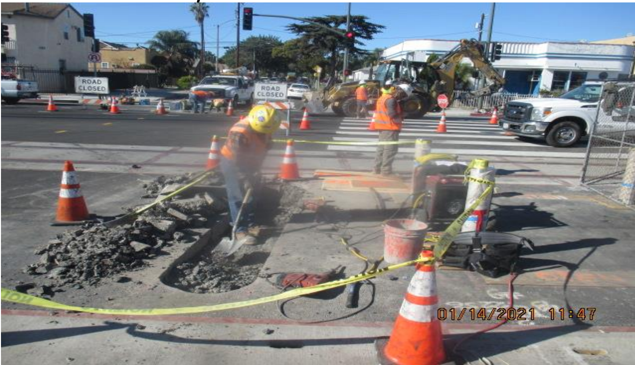
PARK MESA – Excavating for footing of safety curb in front of the stainless steel bollards on the south end crosswalk at 59th St.
