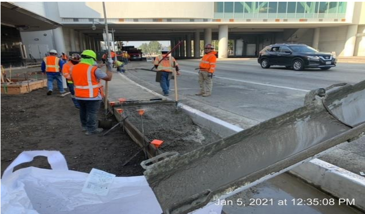
MLK STATION – Placing concrete for new sidewalk installation along the north side of the plaza.
