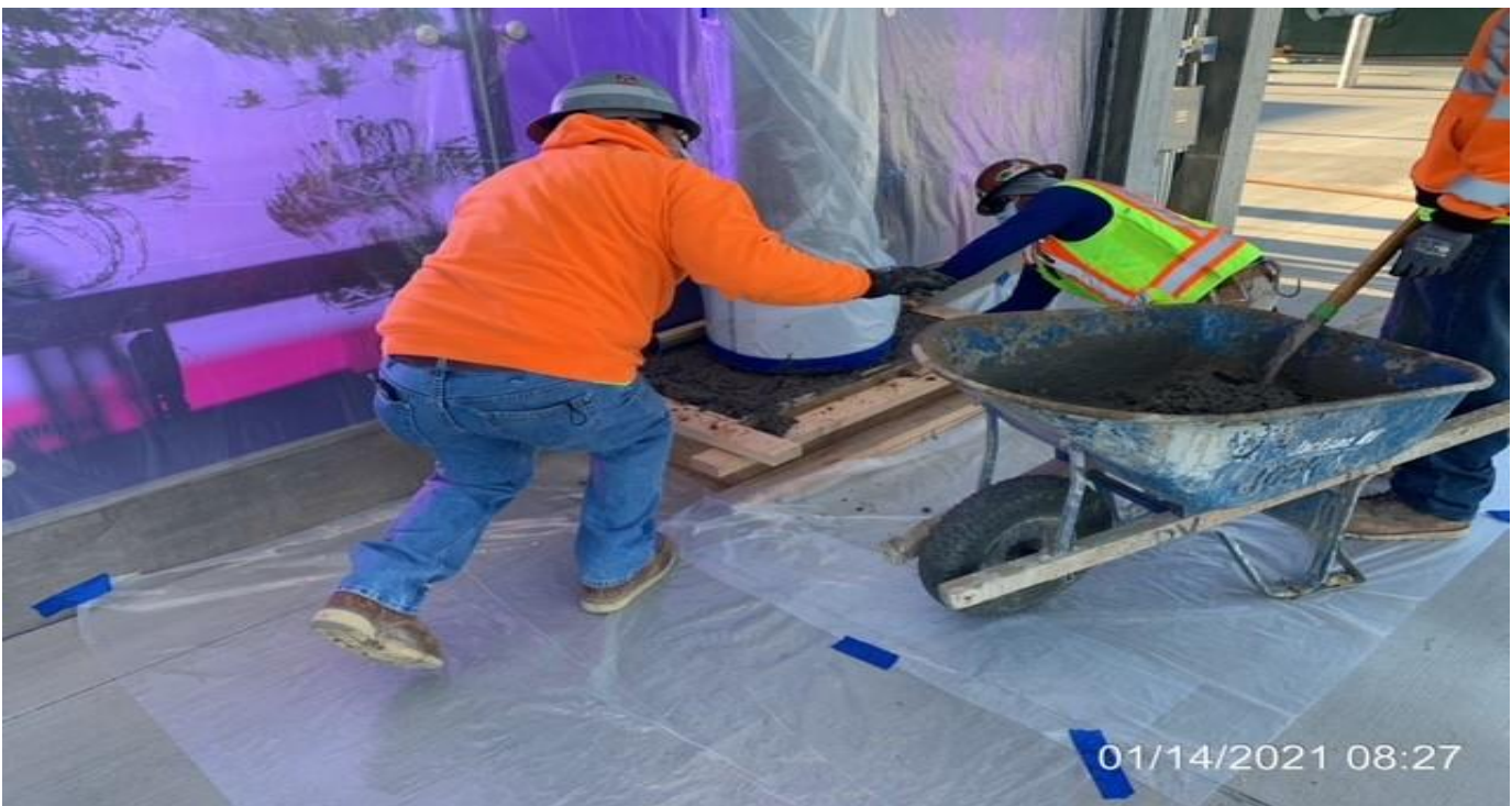
LEIMERT PARK STATION – Placing concrete for the column bases around the main entrance canopy at the plaza.
