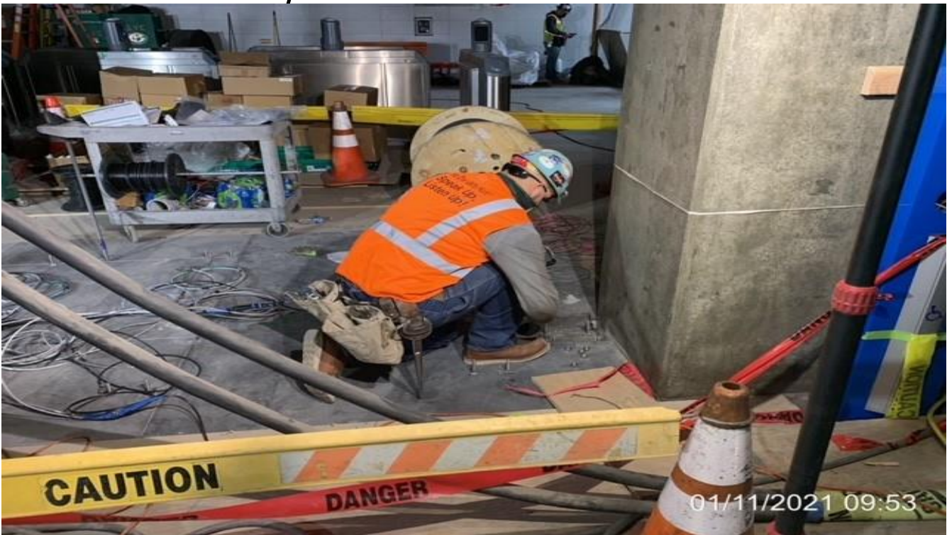
MLK STATION – Anchoring plates for Fare Gate System picket fence posts at the Paid & Free Area.
