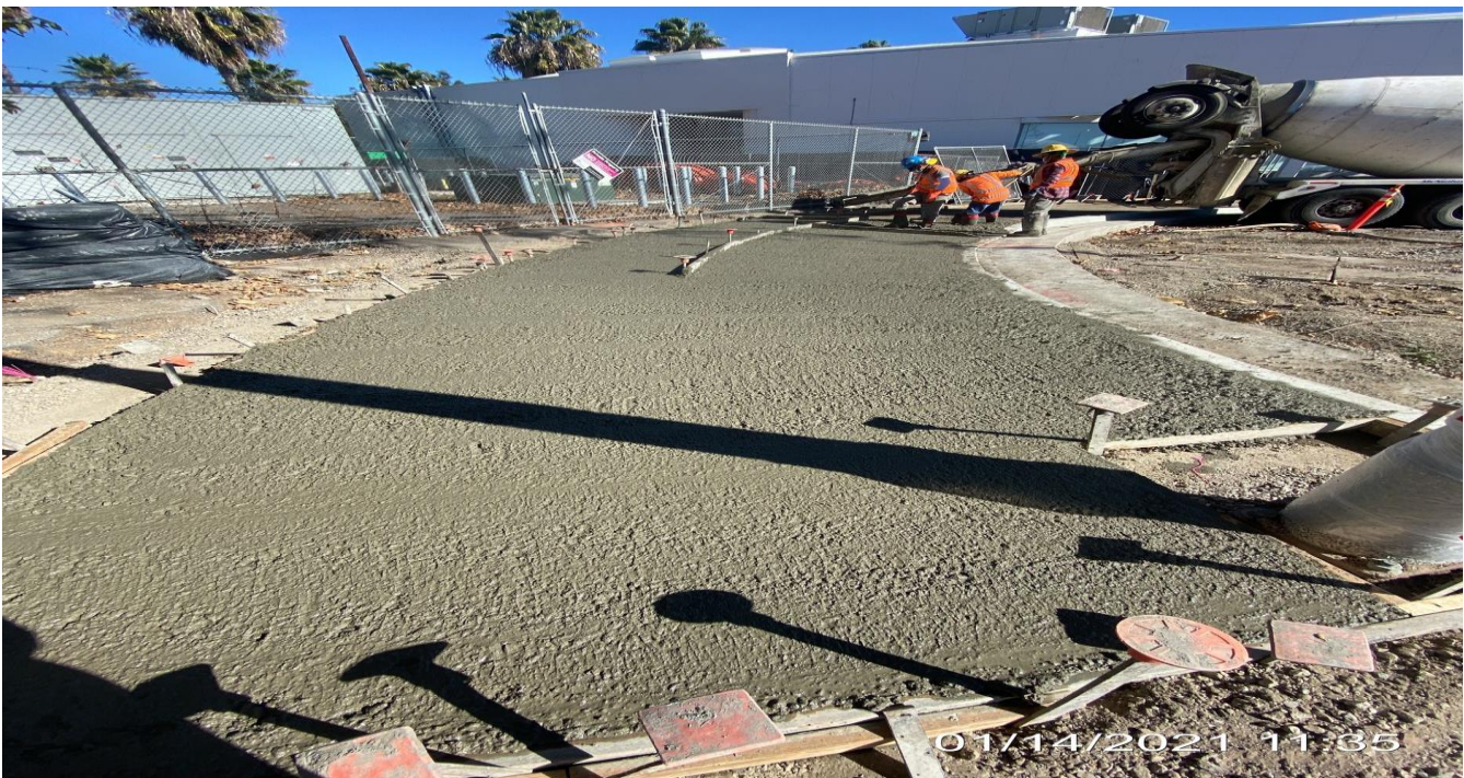
EXPO STATION – Placing concrete for new northbound sidewalk along the Bronson Cul-de-sac.
