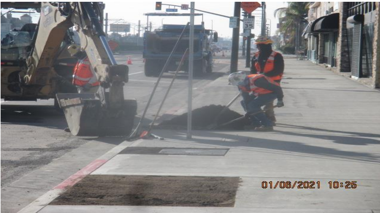
PARK MESA – Continue placing top soil to tree wells along southbound Crenshaw Blvd between 52nd St. and 54th St.
