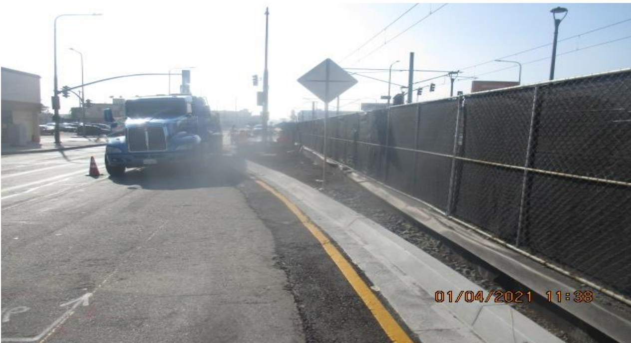
PARK MESA – Continue excavating/grading the northbound median curb on Crenshaw Blvd from 60th St to 59th St.
