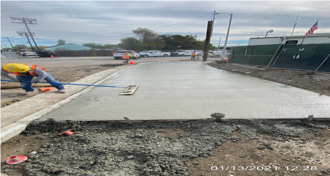
EXPO STATION SITE – Continue placing concrete for new southbound sidewalk along the Bronson Cul-de-sac.
