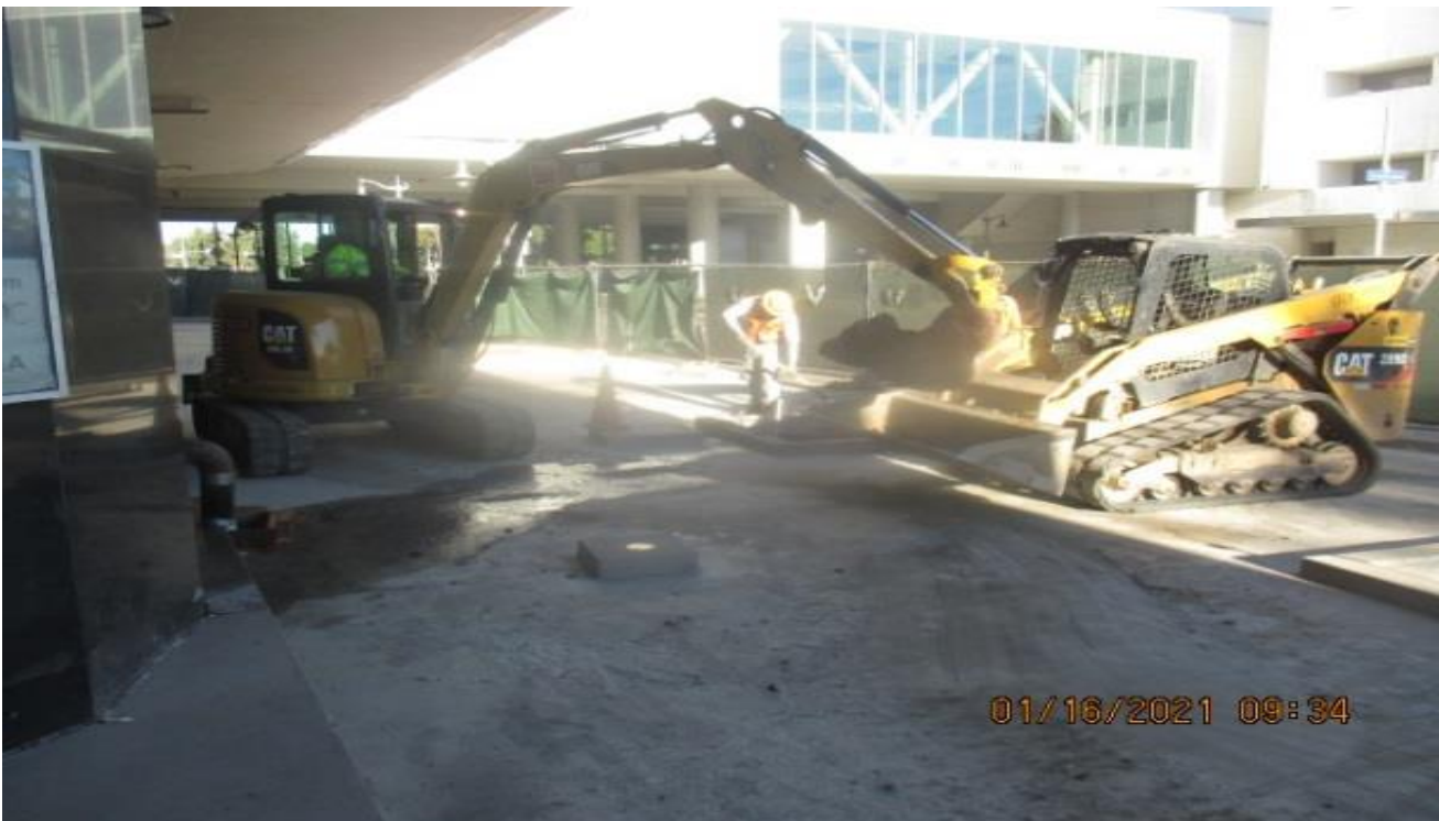
MLK STATION – WSCC crew removing forms from short curb wall along north mall wall.
