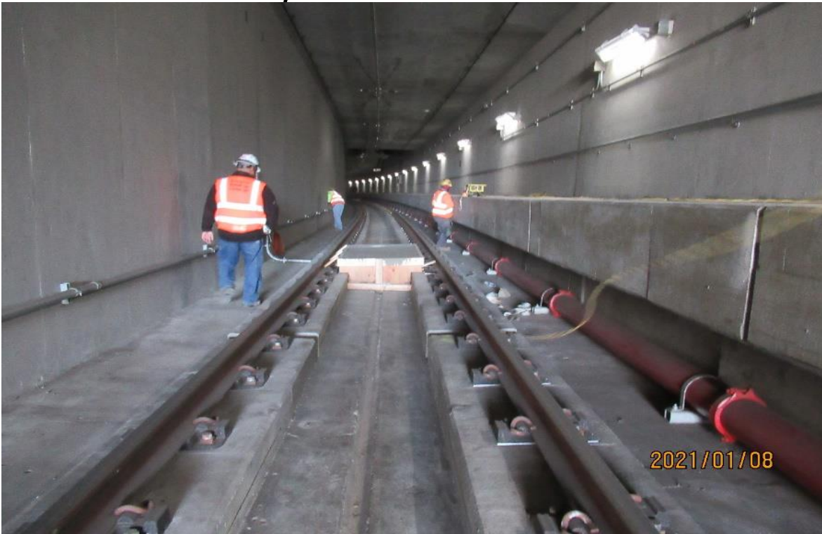
UG4 – WSCC clean-up crew along with WSCC QC inspector in UG4 SB track portal STA 371+10 (looking north).
