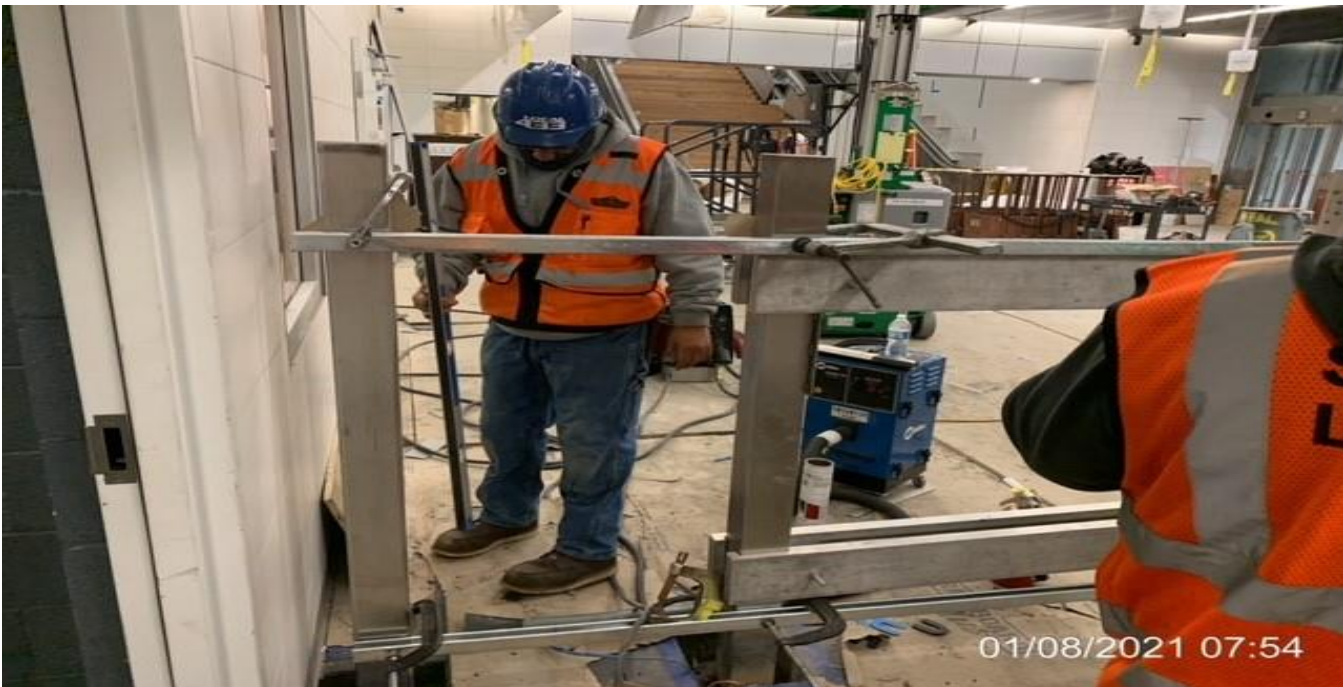
LEIMERT PARK STATION – Installing posts for the Fare Gate picket fence at the Paid & Free Area.
