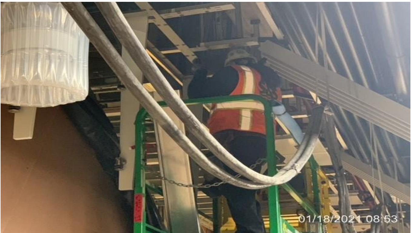
MLK STATION – Installing support framing for stainless steel cladding around the smoke screens of Escalator 4 at the platform.
