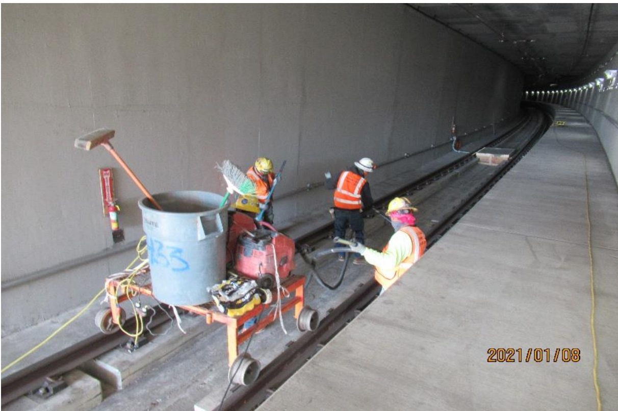
UG4 – WSCC inside portal UG4 SB track STA 371+10 performing general clean-up (housekeeping) looking northwest.
