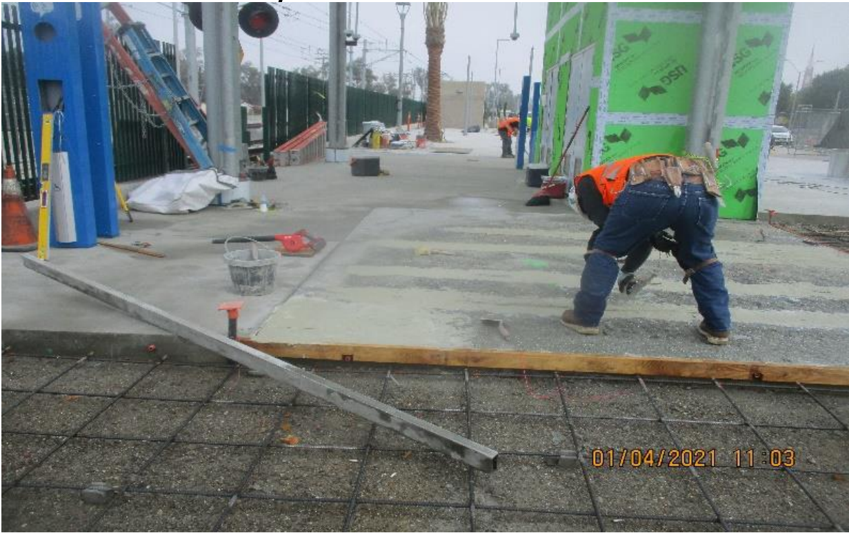
La Brea Station - WSCC Patching and correcting concrete elevation at W/S La Brea Plaza floor.
