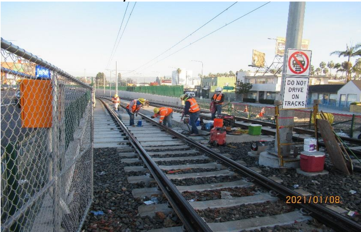
48 th Street – 48th Street SB track WSCC repair crew removing & demoing out loose DF fastener inserts STA 364+48 (looking northeast) Rework for NCR-129 revision-2
