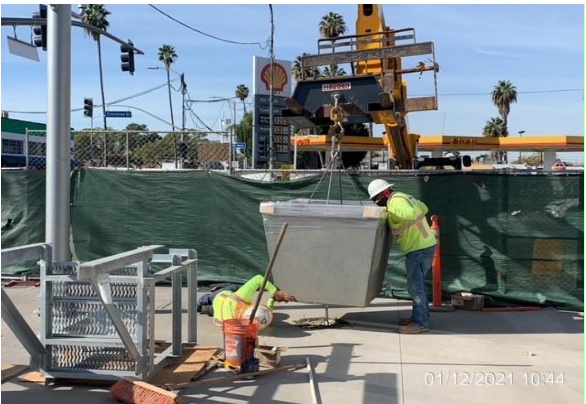
EXPO STATION – Marina Landscaping placing tree pots on west side of station.
