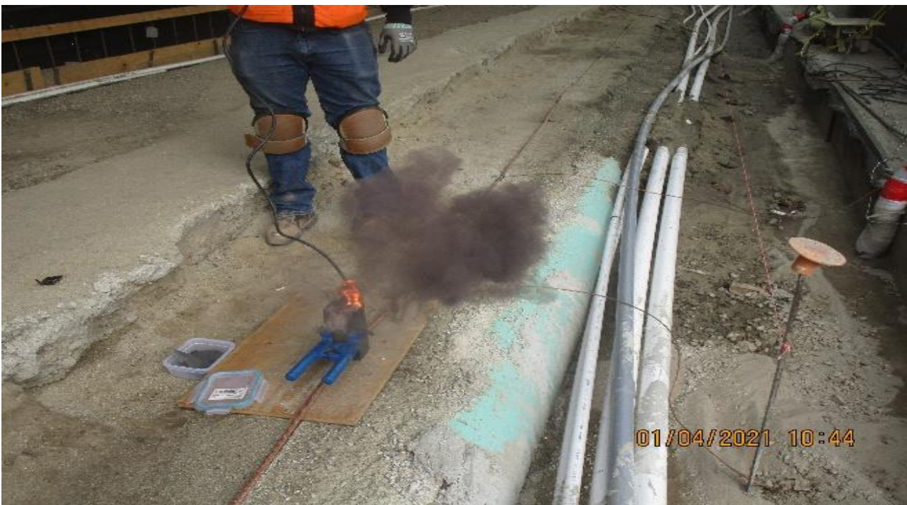
MLK STATION – Continue ground grid installation and bonding of amenities throughout the plaza.
