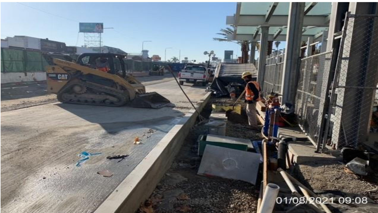
MLK STATION – Backfilling curb on the east side of the main entrance canopy at the plaza.
