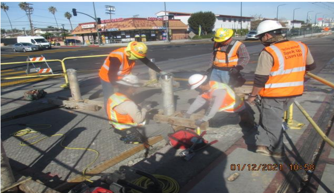
PARK MESA – Installing stainless steel bollards on the north end crosswalk at Slauson Ave.
