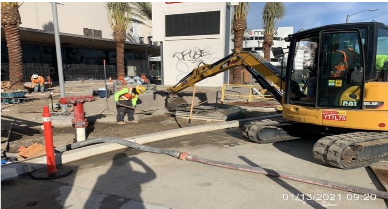
MLK STATION – Grading the entire curb on the east side of the plaza.
