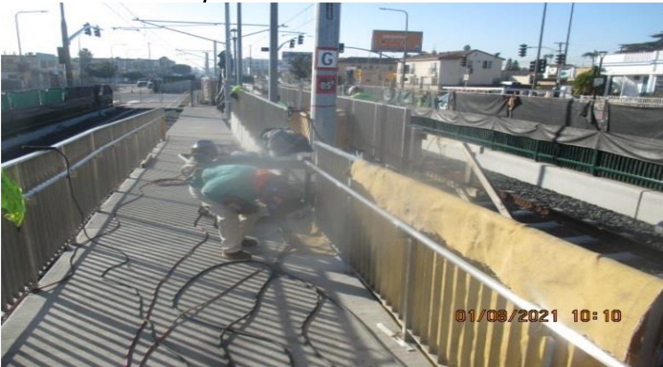
PARK MESA – Grinding and polishing handrail and guardrail finishes at the south entrance walkway ramp.
