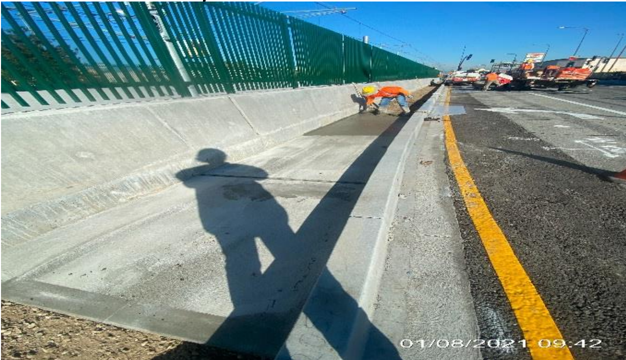
PARK MESA – Placing concrete along the northbound median curb on Crenshaw Blvd from 59th Pl to 59th St.
