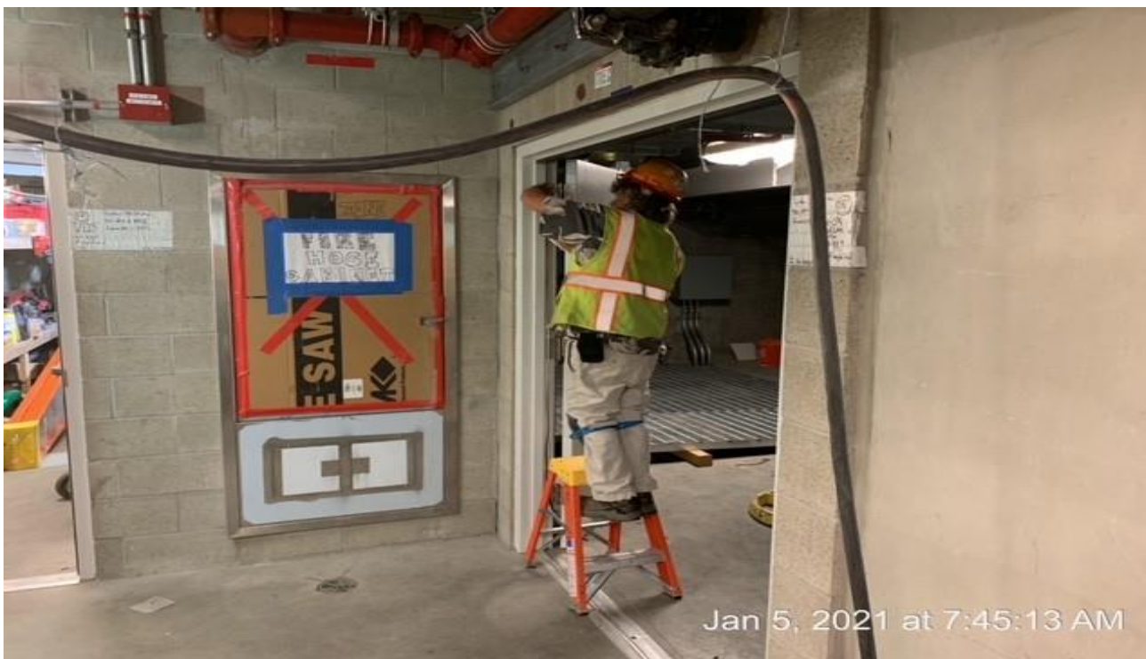
LEIMERT PARK STATION – Installing thresholds, fire smoke seals and closures for doors throughout various room at the concourse.
