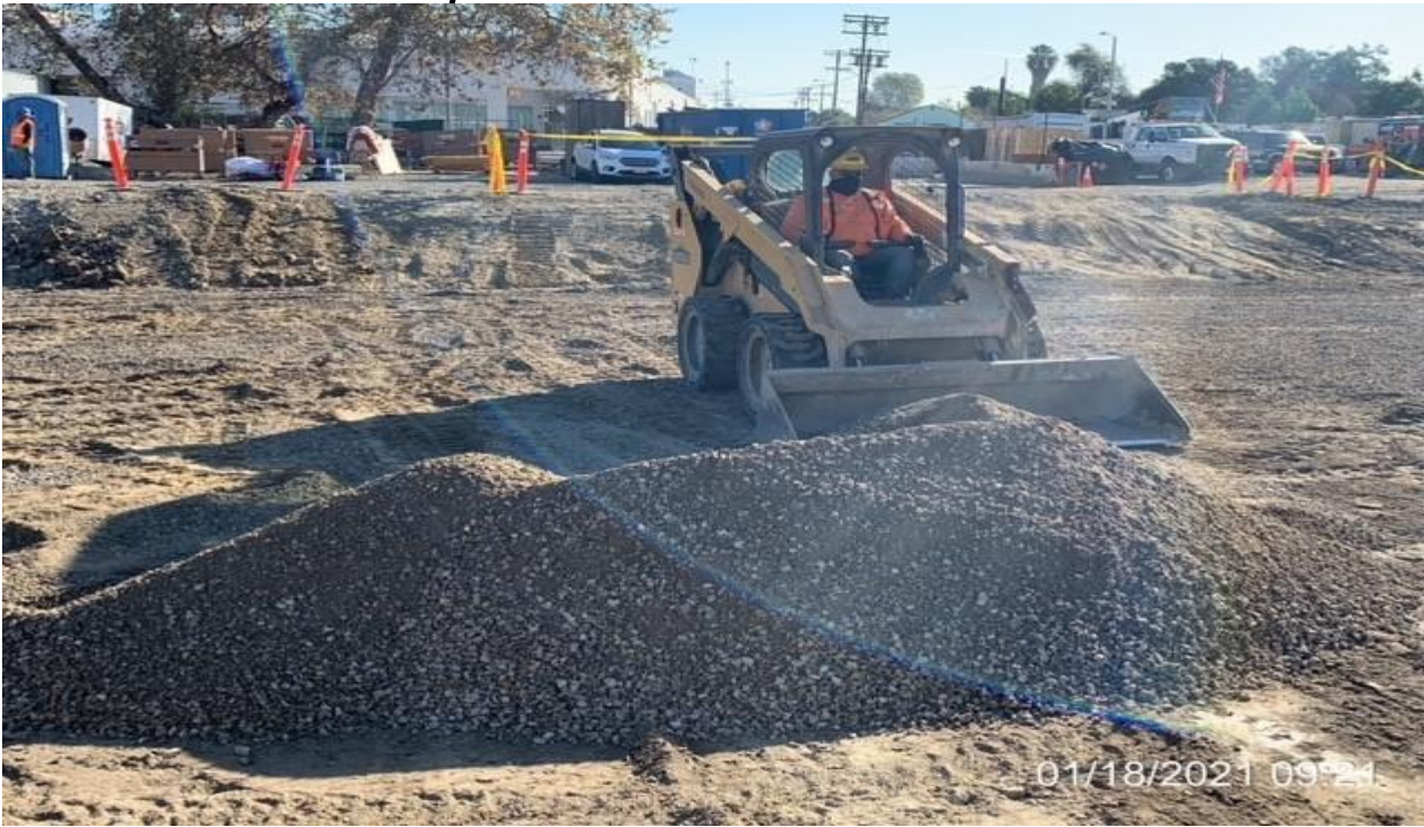
EXPO STATION – Continue rough grading and placing base on the north side of the Park & Ride lot area.
