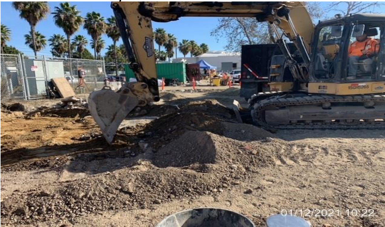
EXPO STATION – Rough grading the west side of the Park & Ride lot area.
