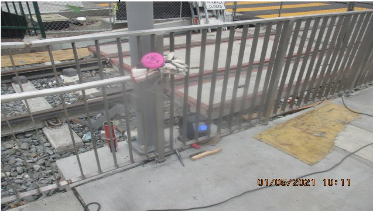
PARK MESA – Continue welding handrails and brackets to the guardrails of the north entrance walkway ramp.
