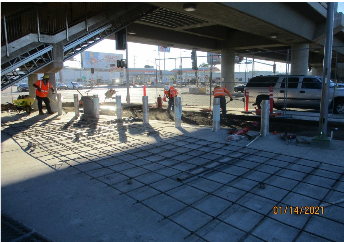
AVIATION/CENTURY- Grading the base for the hardscape at the Aviation Station plaza. Facing SE.
