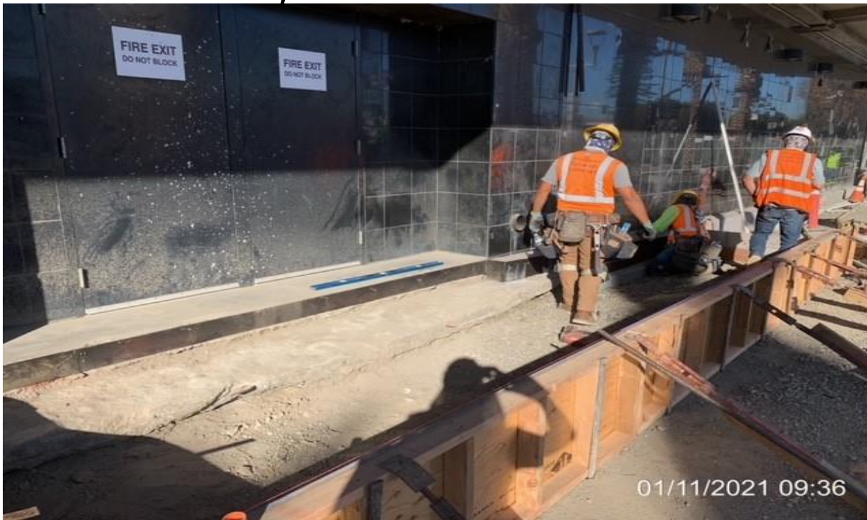
MLK STATION – Building formwork for stair landing installation on the west side of the main entrance canopy at the plaza.
