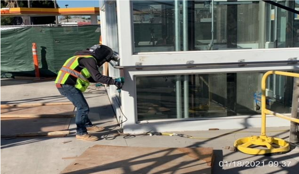
EXPO STATION – Grinding stainless steel handrail finishes of Elevators 1&2 at the plaza.
