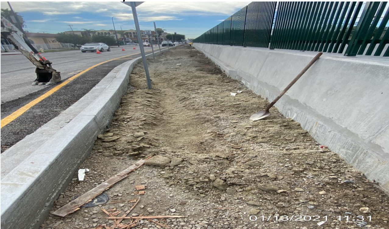
PARK MESA – Prepared for irrigation installation along the northbound median curb on Crenshaw Blvd from 60th St to 59th St.
