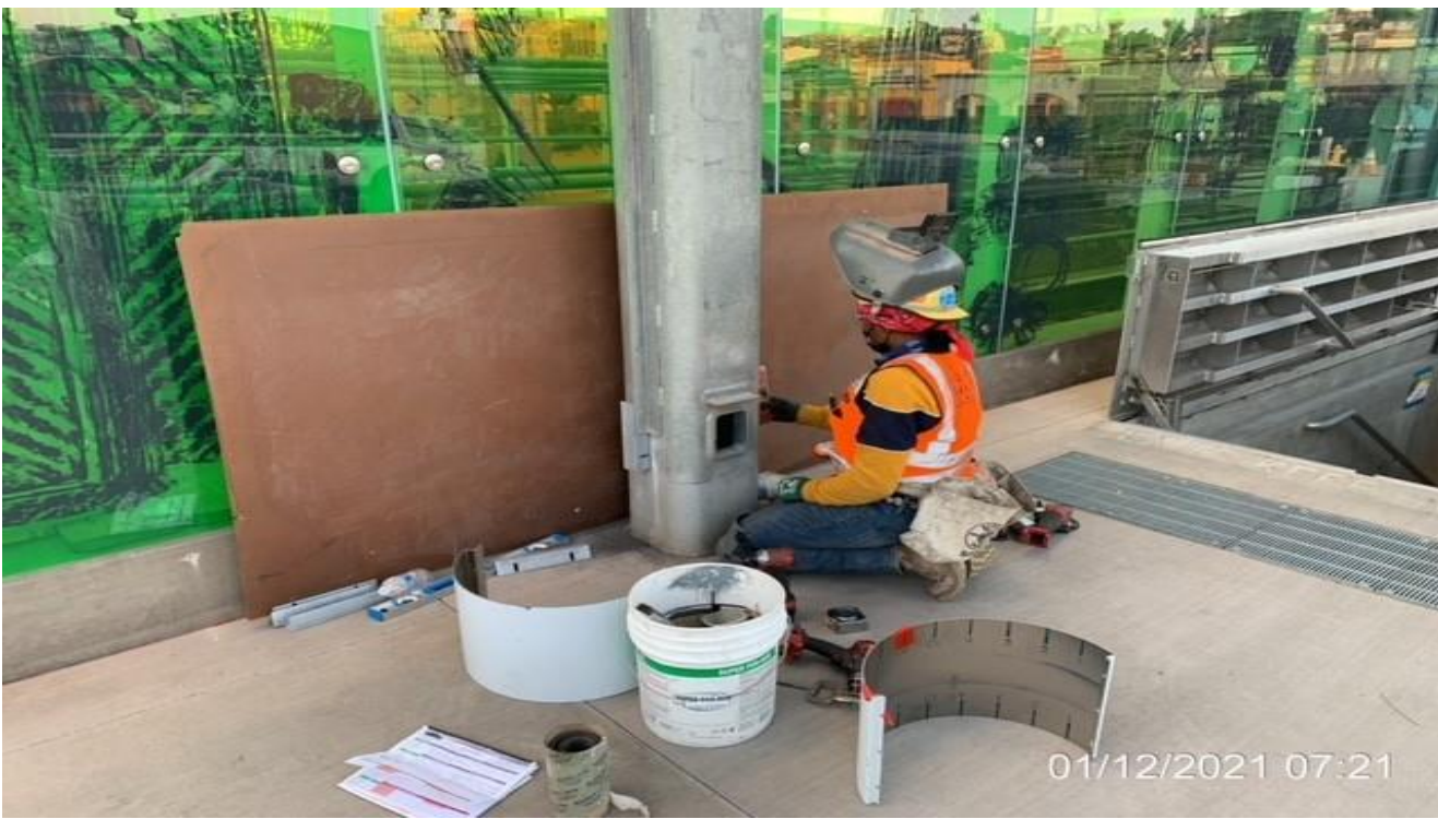
LEIMERT PARK STATION – Installing cladding to column bases around the main entrance canopy at the plaza.
