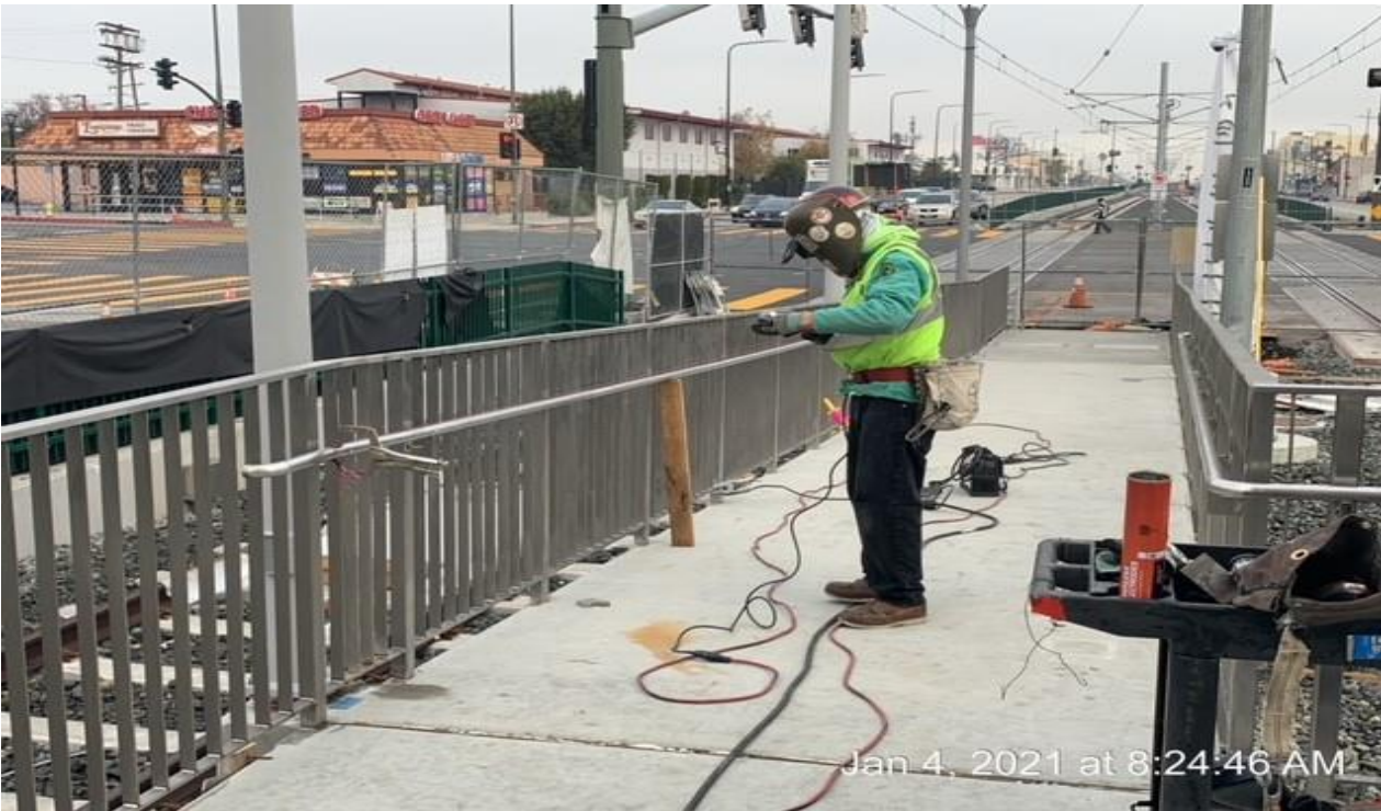
PARK MESA – Welding handrails and brackets to the guardrails of the north entrance walkway ramp.
