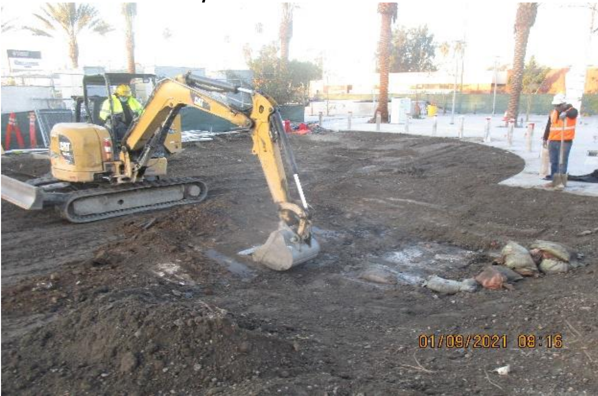
EXPO STATION – continued rough grading slop to drain at beginning of treatment swale #3 & general clean up
