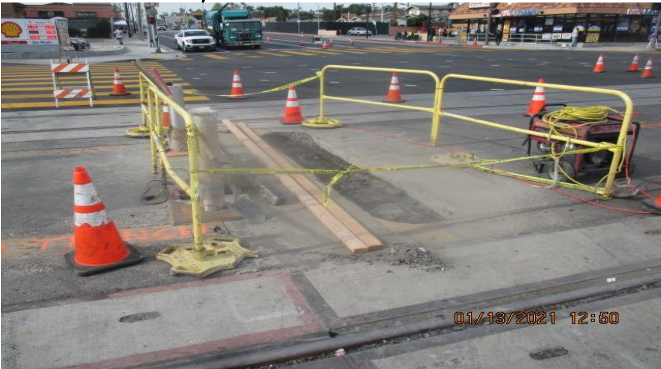
PARK MESA – Excavating for footing of safety curb in front of the stainless steel bollards on the north end crosswalk at Slauson Ave.
