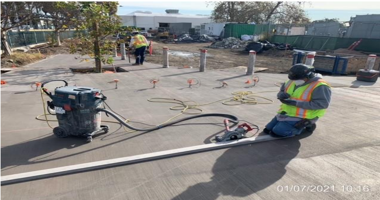
EXPO STATION – Saw cutting control joints to the architectural topping slab at the north side of the plaza.
