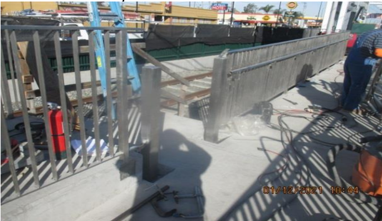
PARK MESA – Installing pedestrian safety gate at the south entrance walkway ramp.
