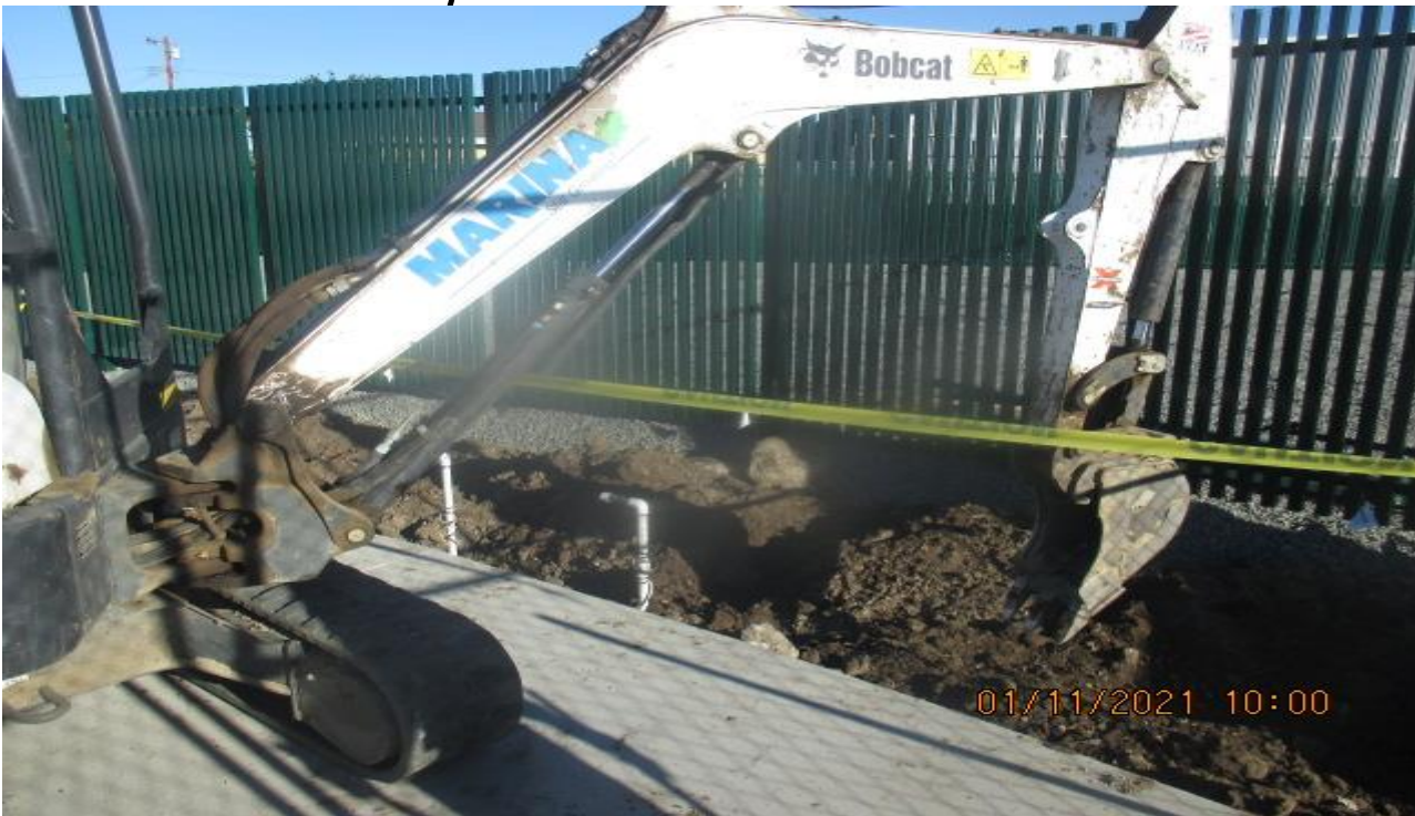
UG3 – Backfilling and installing sprinkler later lines along the Victoria Auxiliary fence on westbound “New Road” and Crenshaw Blvd.
