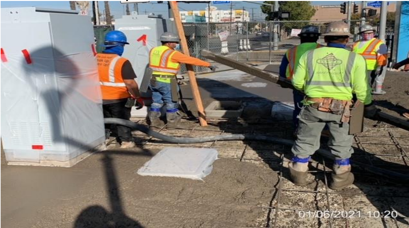
EXPO STATION– Continue placing concrete for the architectural topping slab at the north side of the plaza.
