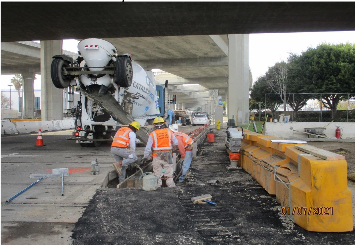
AVIATION/CENTURY- Placing curb and gutter concrete at the NW corner of Aviation and Imperial.
