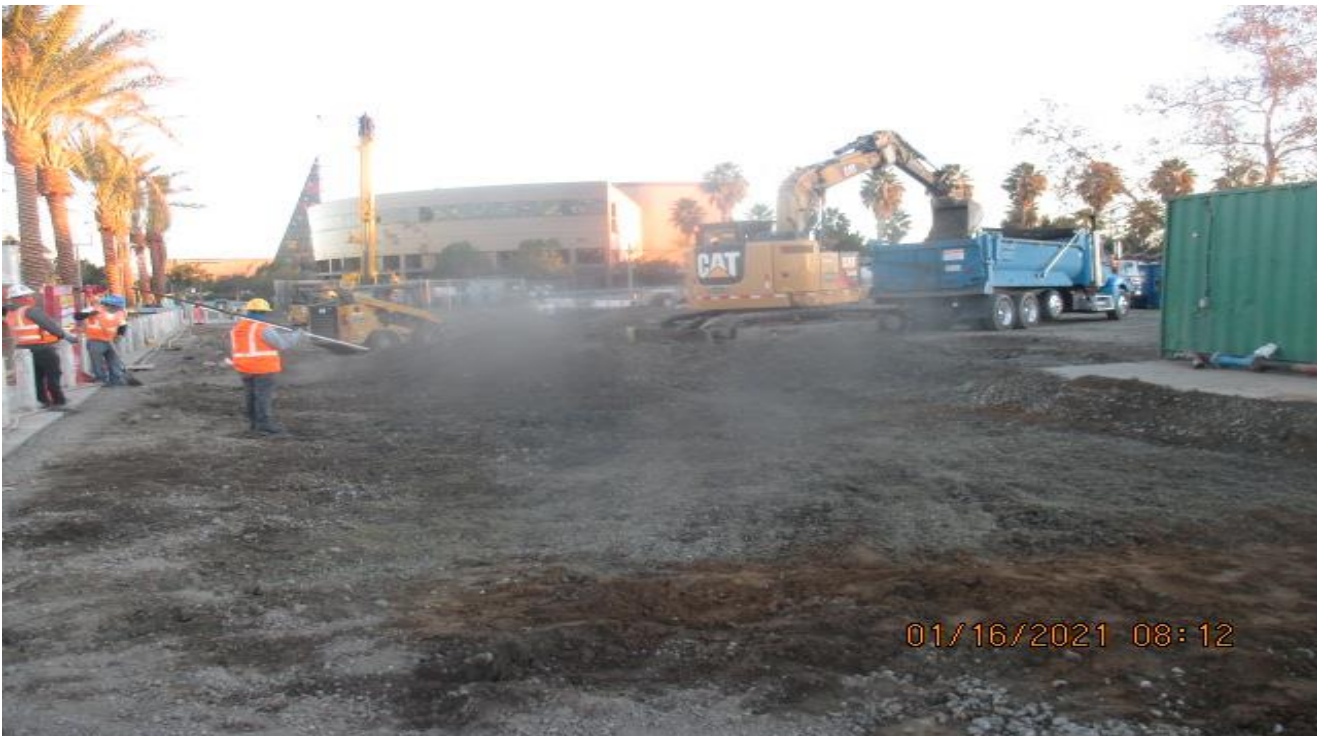
EXPO STATION – Continue rough grading on the west side of the Park & Ride lot area.
