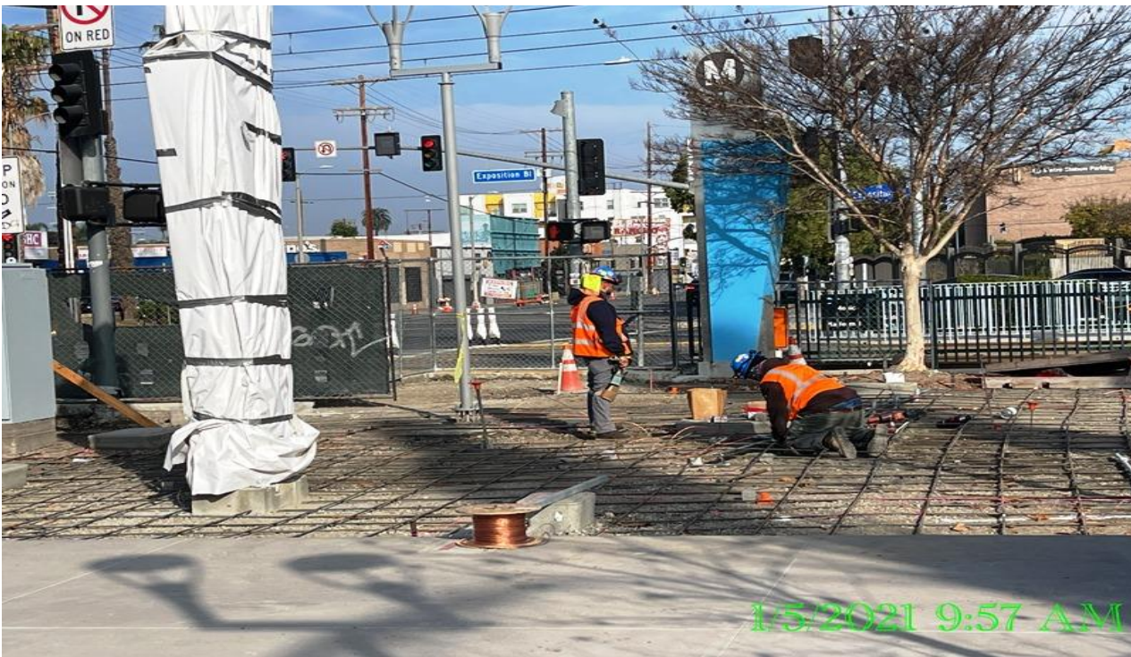
EXPO STATION– Continue ground grid installation at the north side of the plaza.
