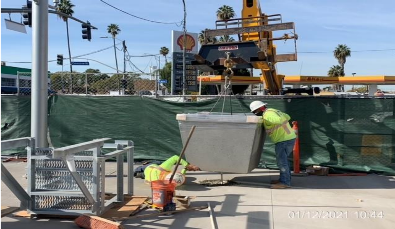
EXPO STATION – Placing planer pots on the west side of the plaza.
