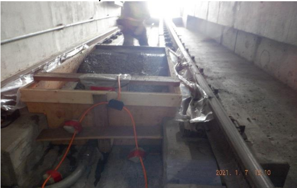
UG4 – STA 372+00 TK#4/NB looking north – UG4 pour PCC traffic loop detector slab.
