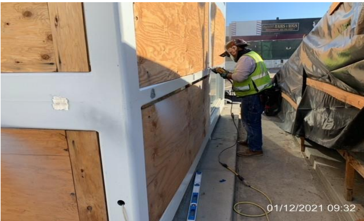
MLK STATION – McMahon installing stainless steel handrail at sides of elevator structure #1 and #2.
