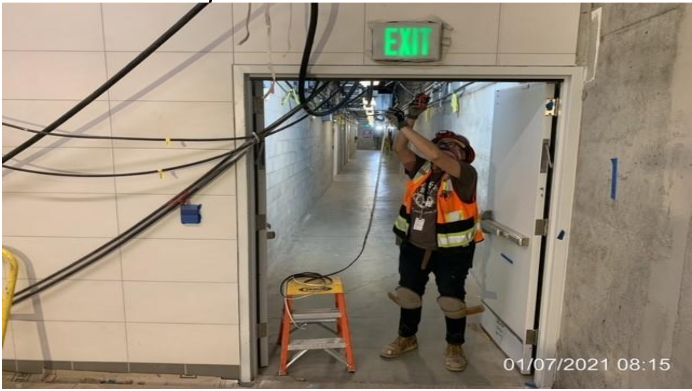
LEIMERT PARK STATION – Continue installing thresholds, fire smoke seals and closures for doors throughout various room at the concourse.
