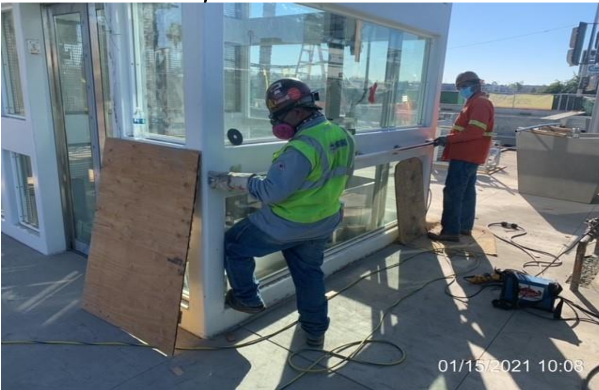
EXPO STATION – McMahon fabricating and installing stainless steel hand rail for structure #1 and #2
