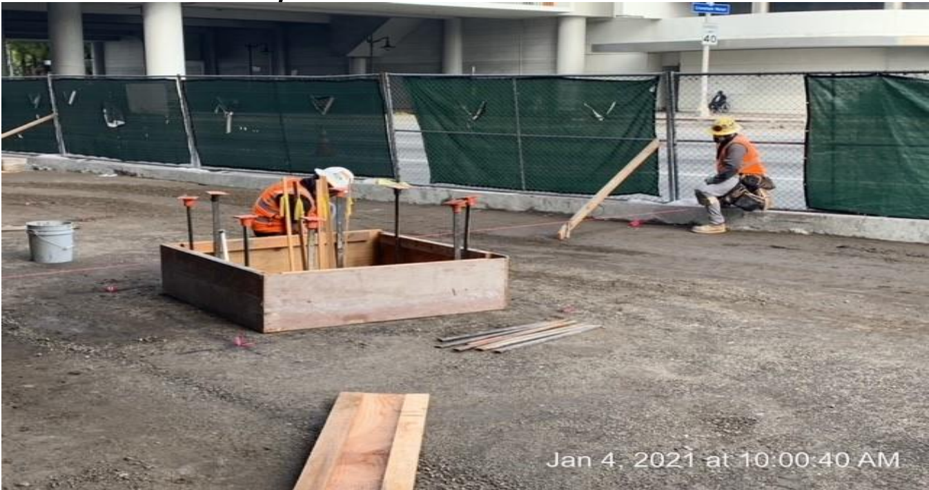
MLK STATION – Continue setting formwork for tree bases at the far northwest area of the plaza.
