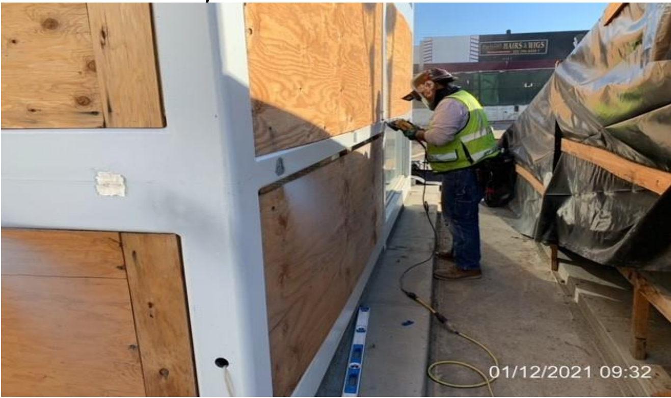
MLK STATION – Installing stainless steel handrails to the sides of Elevators 1&2 at the plaza.
