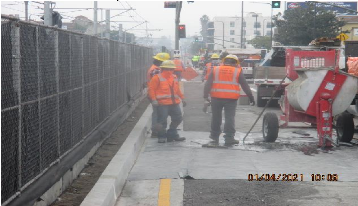
PARK MESA – Mixing and placing mortar base for cobble installation on the southbound median curb on Crenshaw Blvd from 59th St to 58th Pl.
