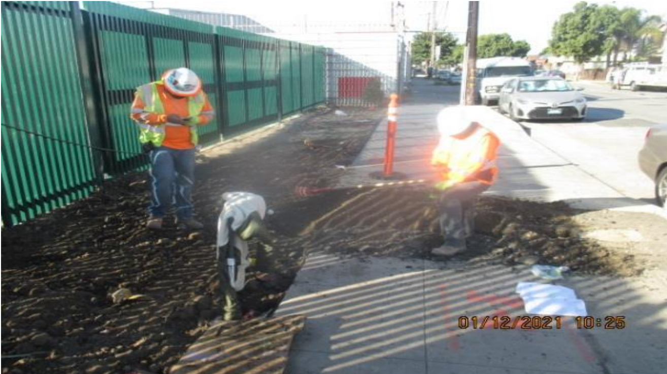
UG3 – Backfilling and installing sprinkler later lines along the Victoria Auxiliary fence on eastbound 67th St and Crenshaw Blvd.
