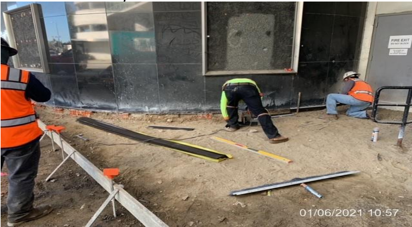
MLK STATION – Continue expansion board installation along the north side curb of the Mall in preparation for concrete placement.
