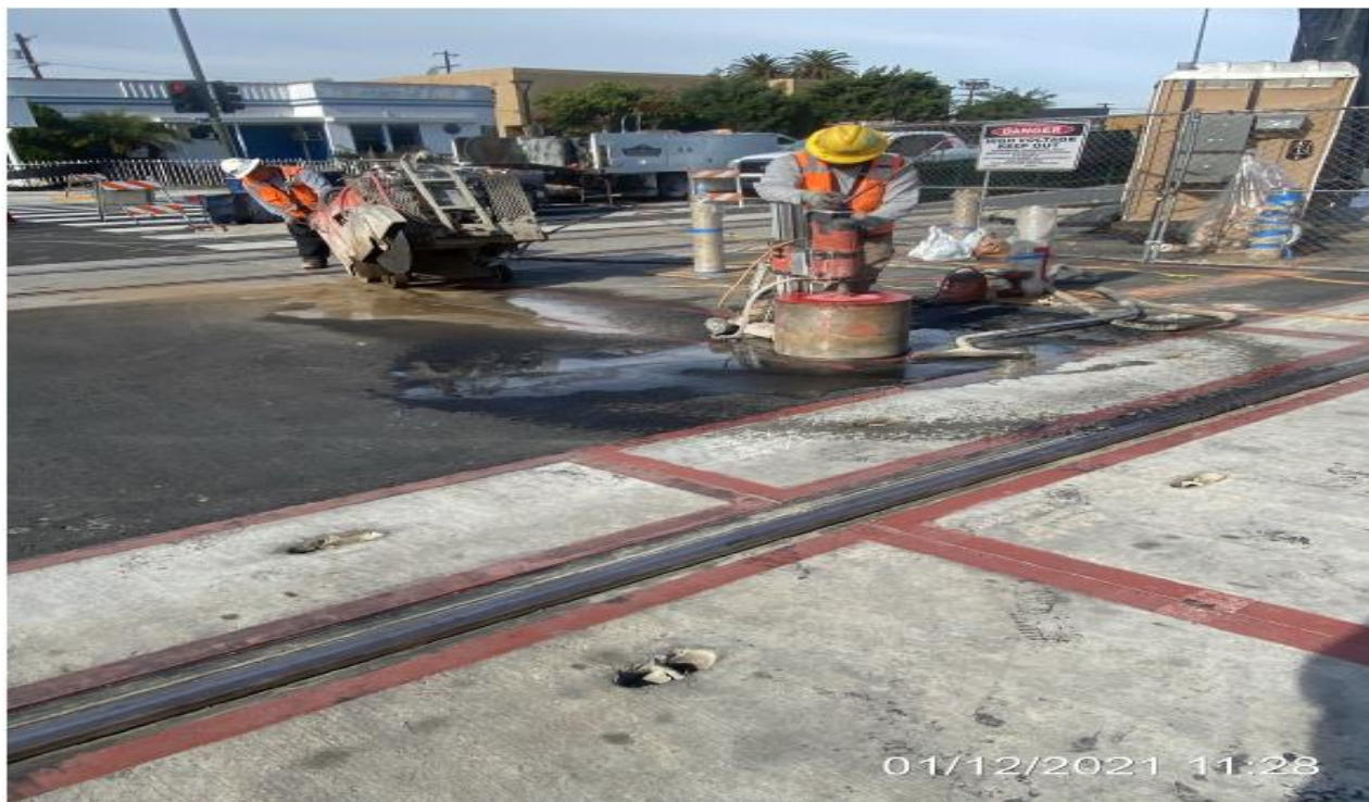
PARK MESA – Saw cutting pavement in preparation of stainless steel bollard installation on the south end crosswalk at 59th St.
