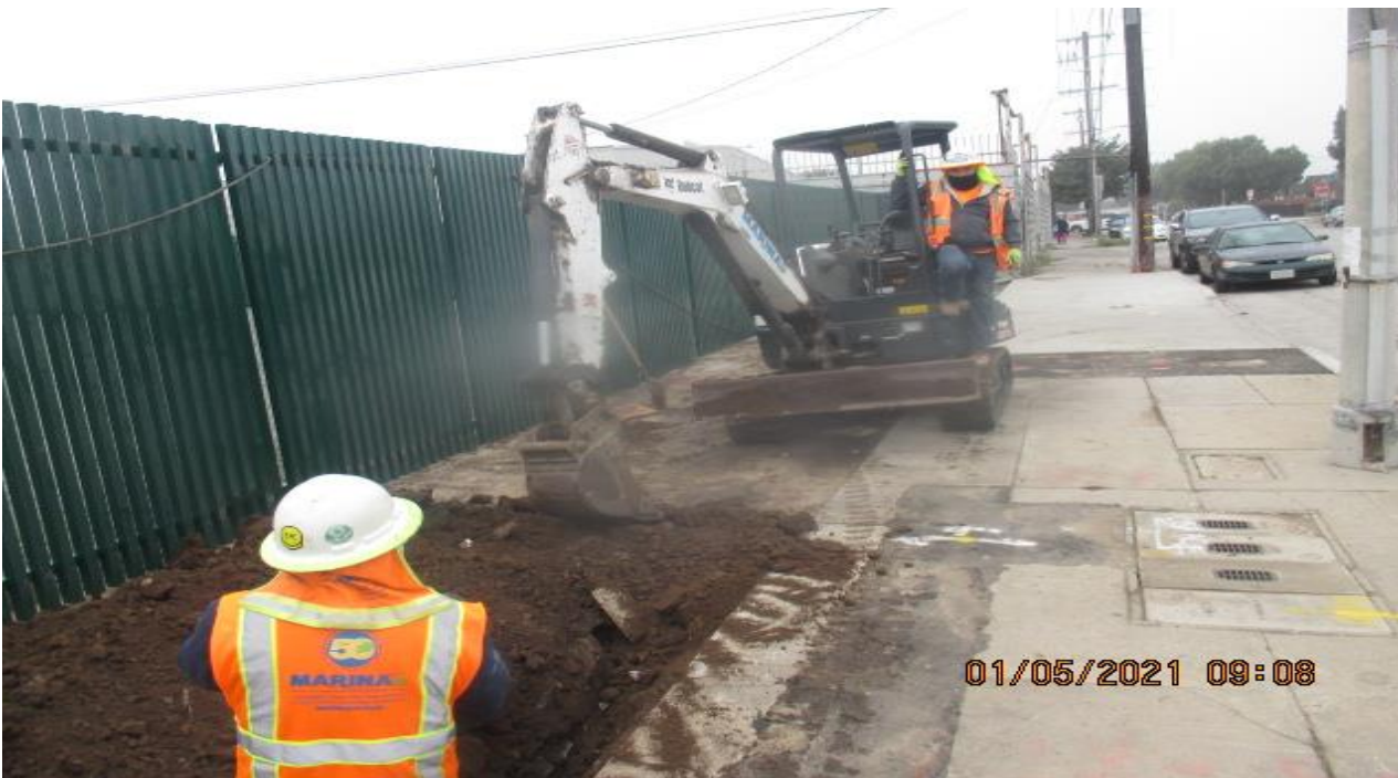
UG3 – Excavating/trenching for main irrigation line along the Victoria Auxiliary fence on eastbound 67th St and Crenshaw Blvd.
