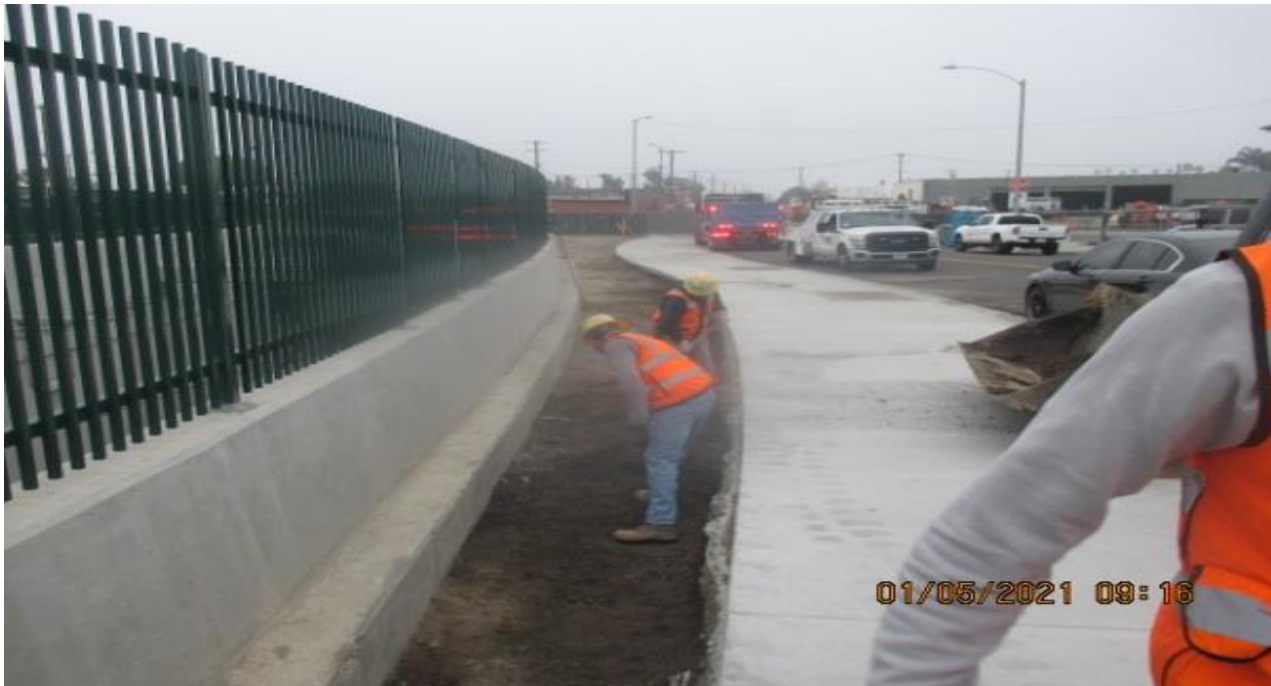
UG3 – Excavating/grading between the back of sidewalk and northbound barrier wall on westbound “New Road” and Crenshaw Blvd.
