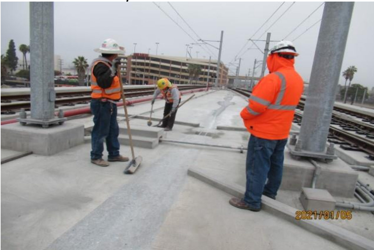
AVIATION/CENTURY- WSCC crew on Century/Aviation bridge performing cleanup work (looking north) Rework for Structure
