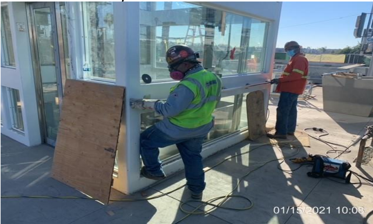
EXPO STATION – Installing stainless steel handrails to the side of Elevators 1&2 at the plaza.
