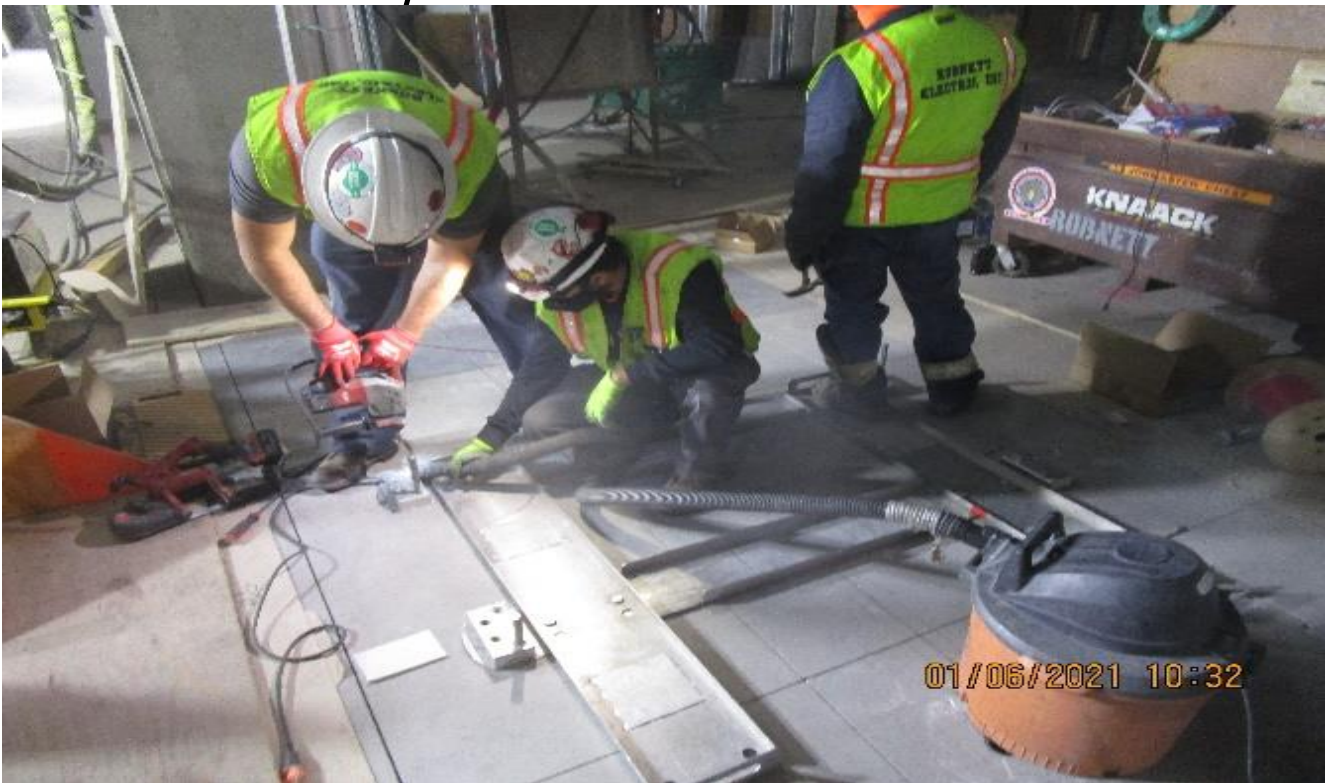
MLK STATION – Continue layout and coring through the walker ducts in preparation for the turnstile fare gate system installation at the Paid & Free Area.
