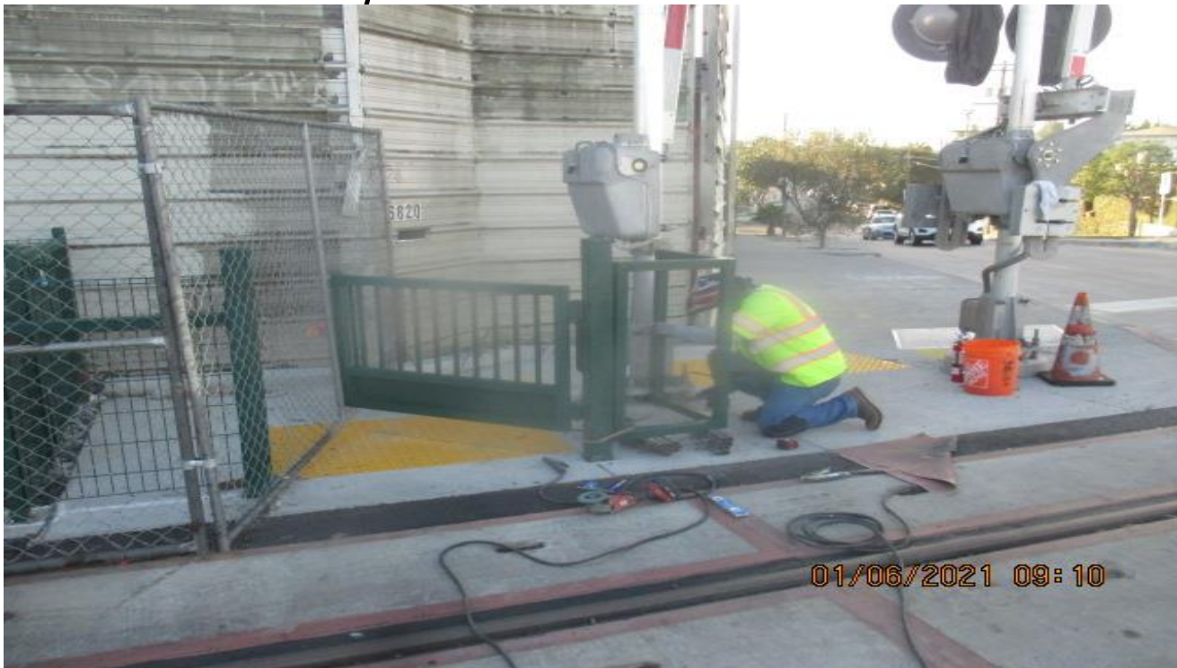
UG3 – Installing pedestrian safety barriers at the track crosswalks of Brynhurst Ave. on both north and southbound side.
