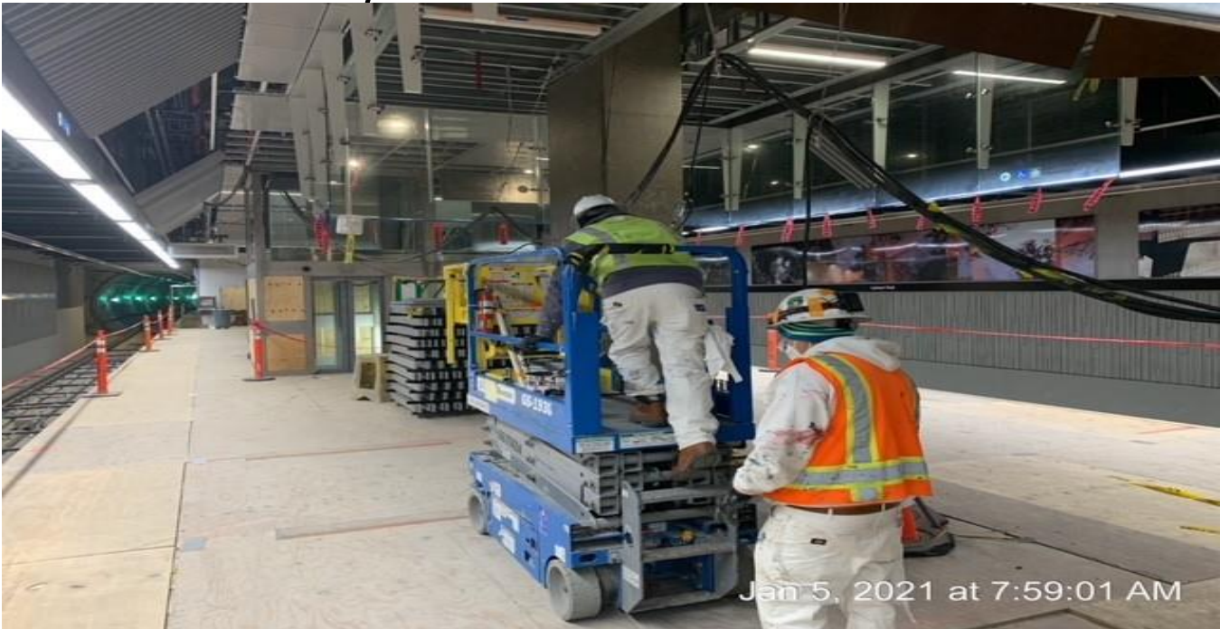
LEIMERT PARK STATION – Preparing to apply primer paint coat to conduits and brackets behind the diagonal screen ceiling panels along the north and southbound side of the platform.
