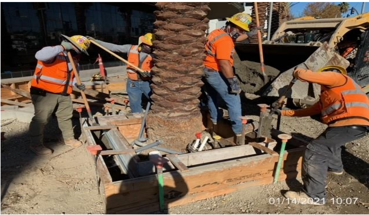
MLK STATION – Resume concrete placement of tree well curbs at the plaza.
