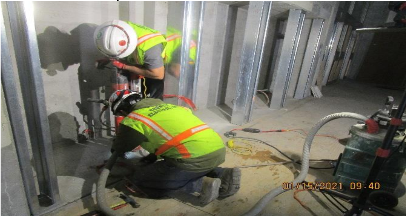
MLK STATION – Performing layout and coring for ticket vending machine installation at the Free Area.
