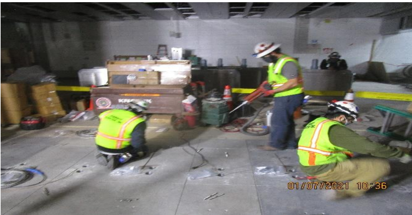
MLK STATION – Continue layout and coring through the walker ducts in preparation for the turnstile fare gate system installation at the Paid & Free Area.
