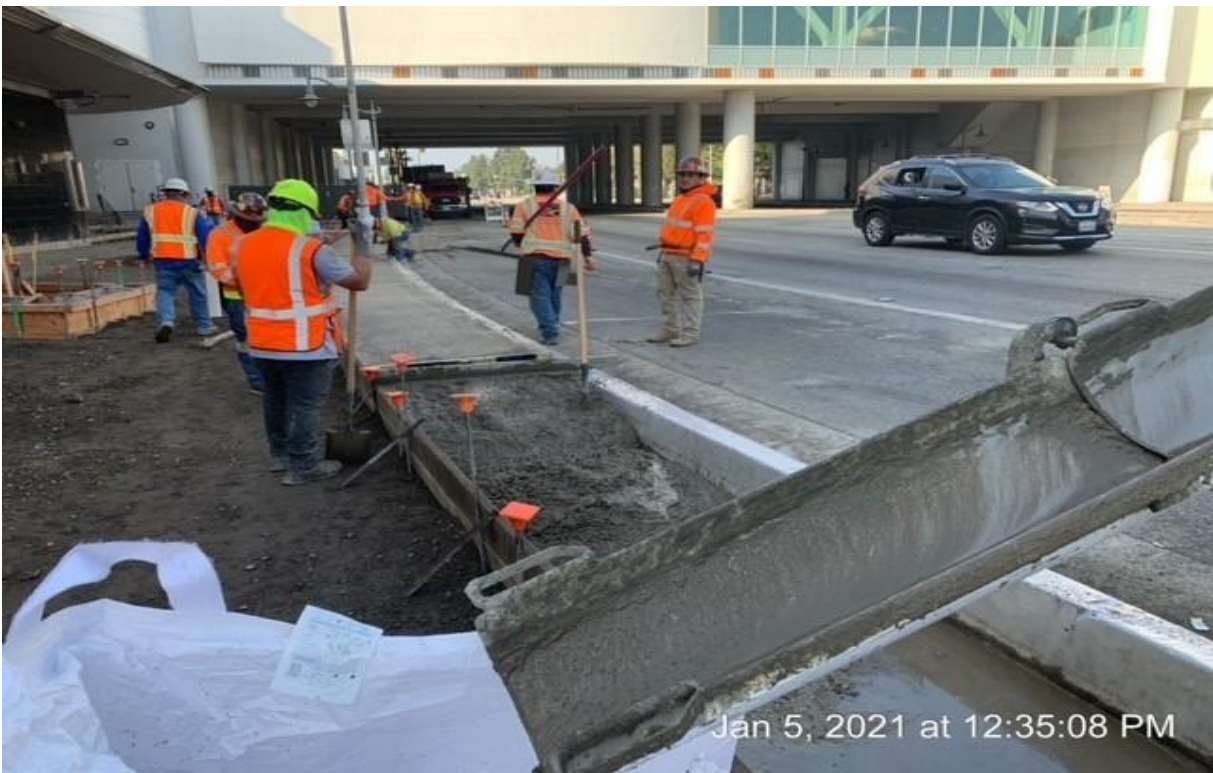
MLK STATION – Griffith placing concrete for sidewalk at north end of station.
