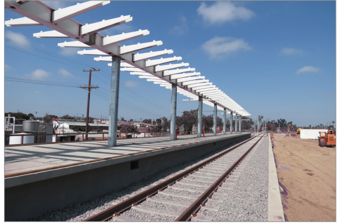
Long Range Planning Projects Station under construction along Crenshaw Line, one of many new transit stations funded by Measure M (Los Angeles)
