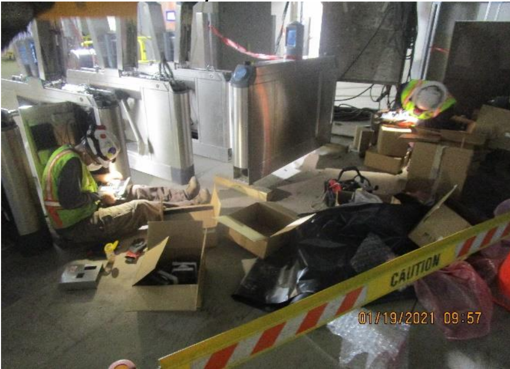
MLK STATION – Performing electrical work to the fare gate turnstiles at the Paid & Free Area.
