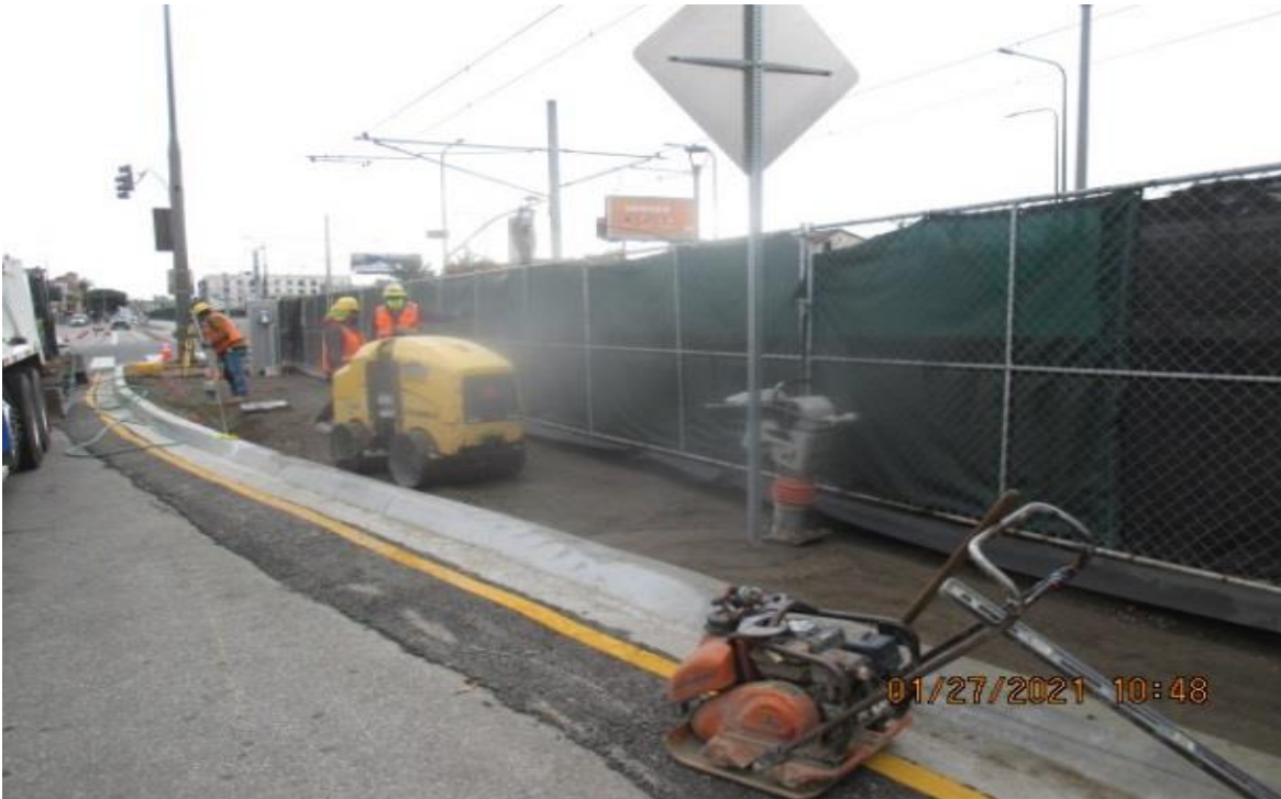
PARK MESA – Backfilling and compacting to grade in preparation for cobble installation along the north and southbound median curbs.
