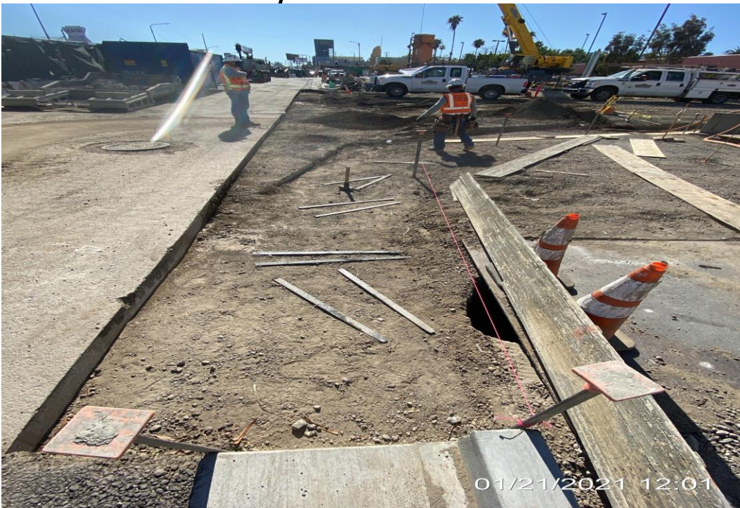
MLK STATION – Placing formwork for new curb and gutter installation along the access road south of the plaza.
