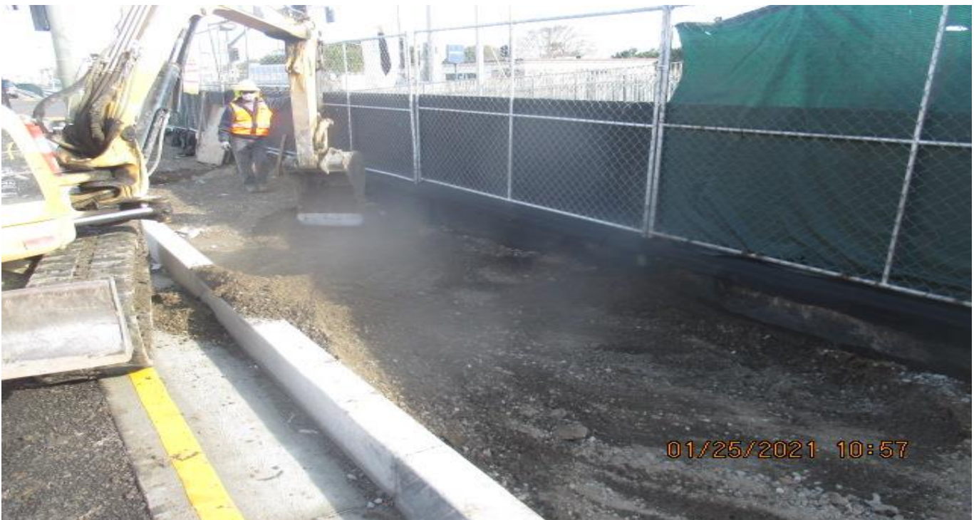
PARK MESA – Excavating for swale channel installation along the southbound median curb on Crenshaw Blvd from Slauson Ave to 59th St.
