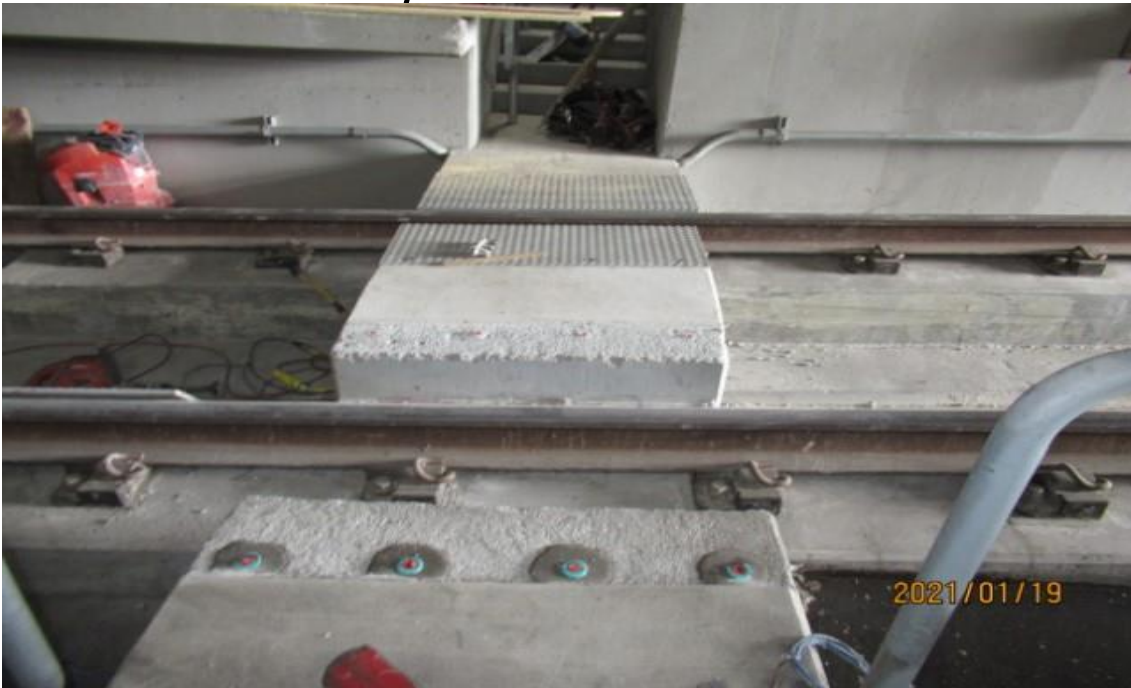
UG4 – UG4 NB track near portal STA 371+25 WSCC on-going work on emergency walkway plates for matching TOR elevations (looking east)
