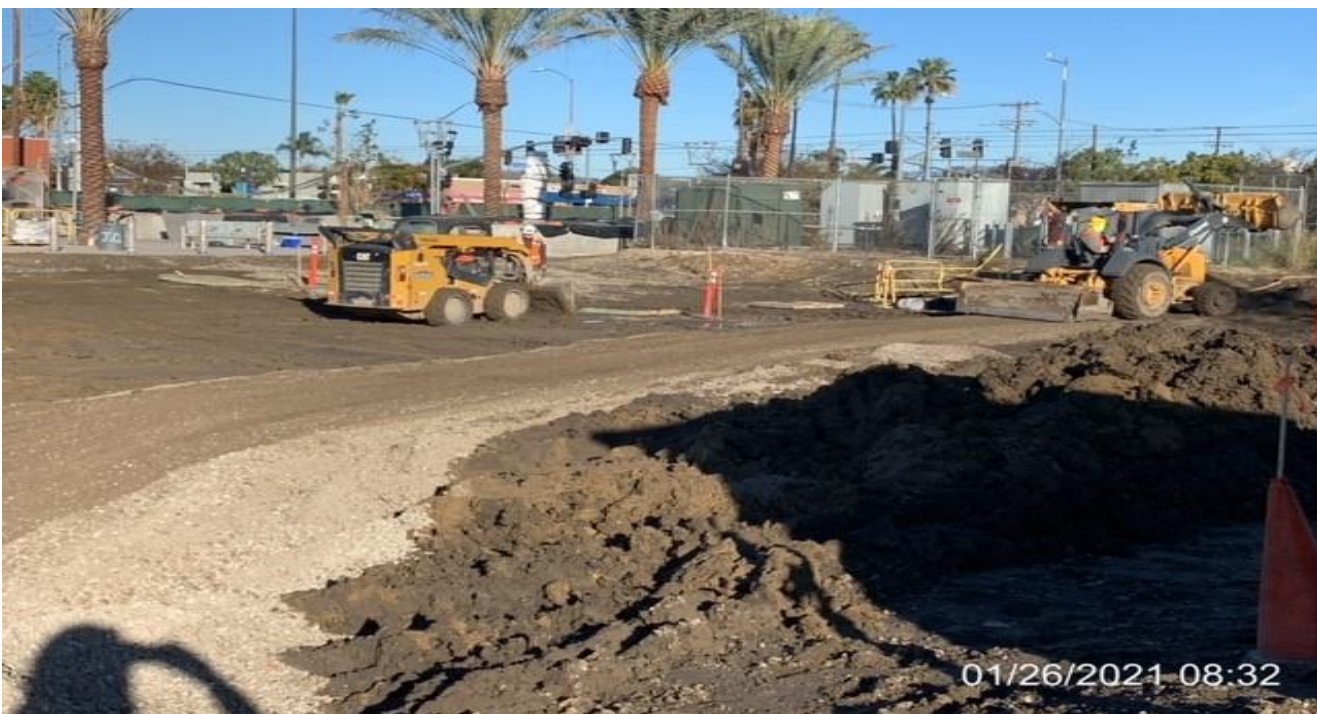
EXPO STATION– Placing base and grading throughout the entire Park & Ride lot area.
