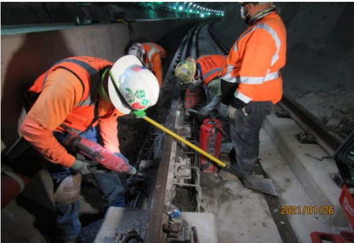
UG4 – WSCC using electrical jack hammers to control demo out plinth 160 in UG4 NB track (looking north) Rework
