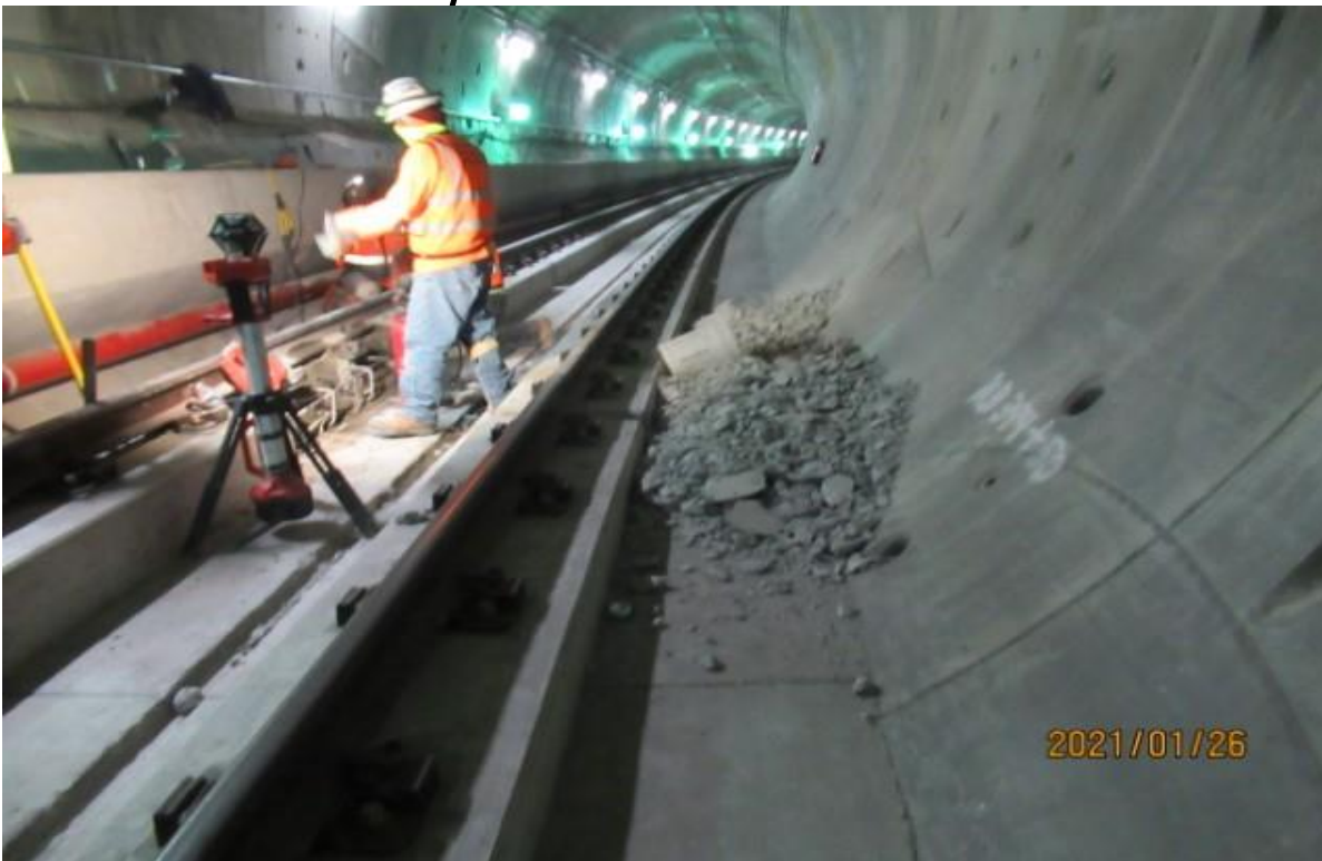
UG4 – UG4 NB track at STA 394+55 WSCC plinth 160 left side partial demo (looking north) Rework
