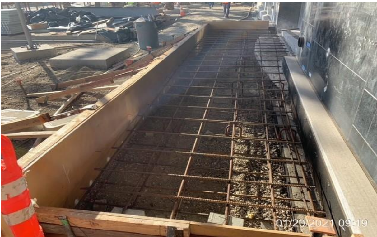
MLK STATION – Installed rebar for stair landing and ADA ramp adjacent to the west side of main entrance at the plaza.
