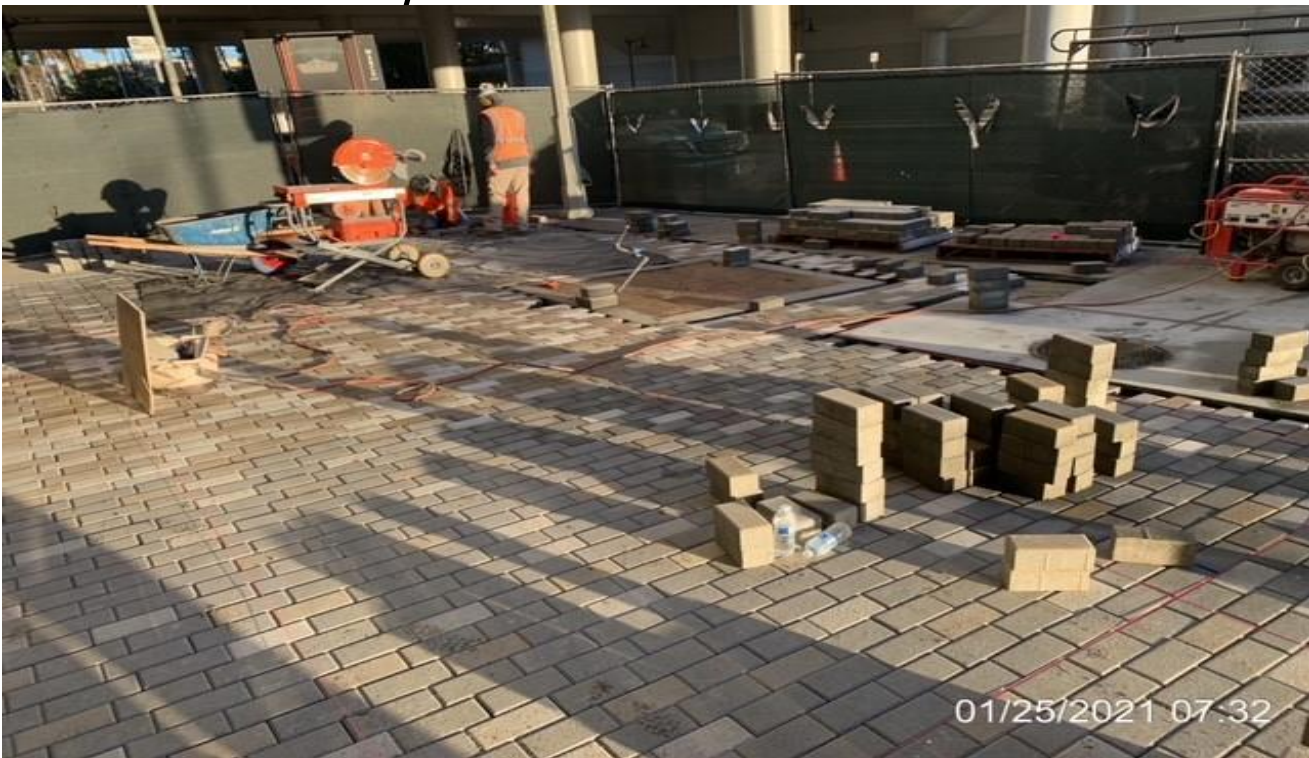
MLK STATION – Continue laying bedding sand and installing brick pavers at the far northwest plaza area.
