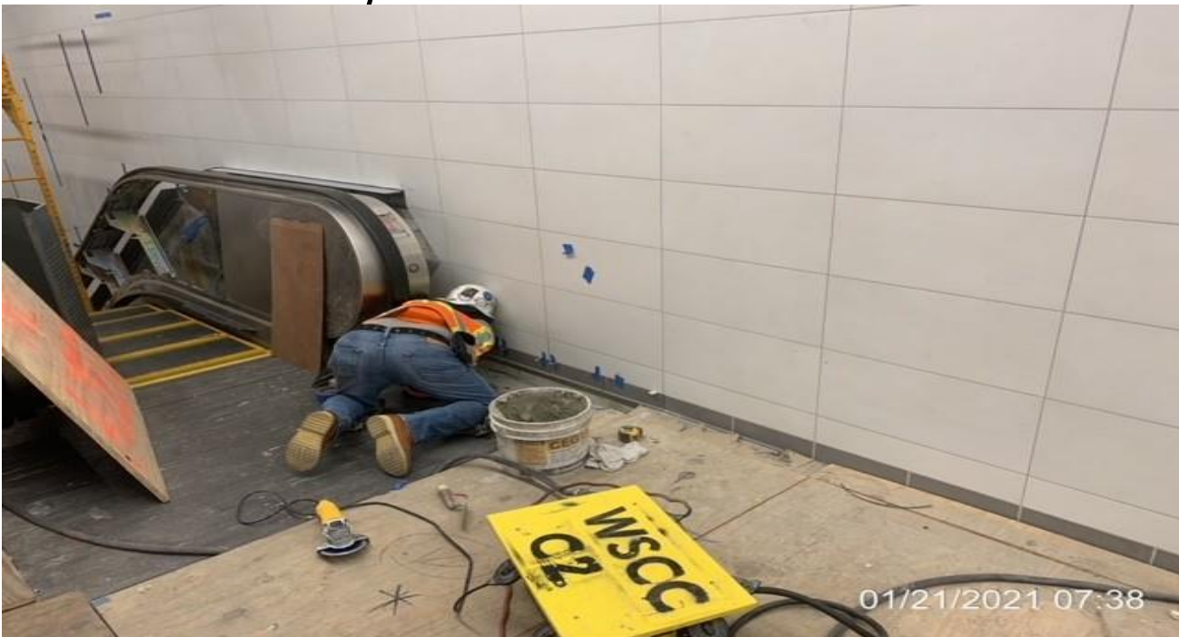
LEIMERT PARK STATION – Continue installation of remaining tiles at base cove locations from intermediate landing to concourse.
