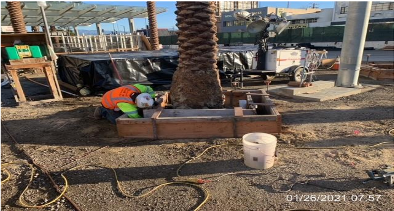
MLK STATION – Building formwork for tree wells bases at the south end of the plaza.
