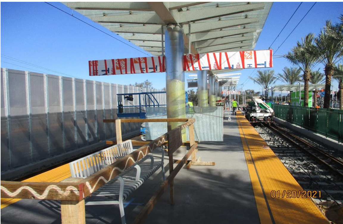
La Brea Station - Glass replacement for the La Brea Station platform canopy.
