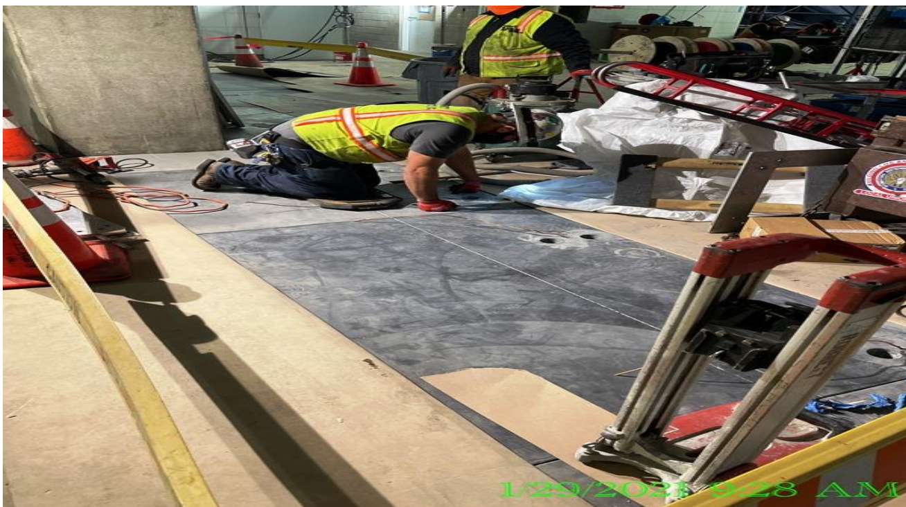
EXPO STATION– Continue performing layout in preparation for fare gate turnstile installation at the Paid & Free Area.
