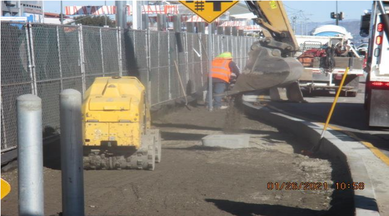
PARK MESA – Placing mortar in preparation for cobble installation along the north and southbound median curbs.
