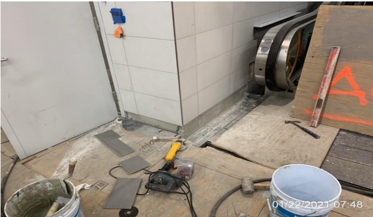
LEIMERT PARK STATION – Continue installation of remaining tiles at base cove locations from intermediate landing to concourse.
