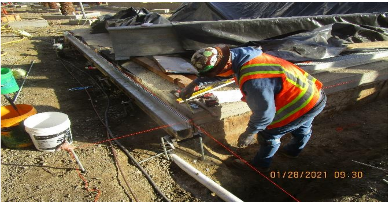
MLK STATION – Installing precast channel drains and HDPE pipe for storm drain tie-in along the west side of the plaza.
