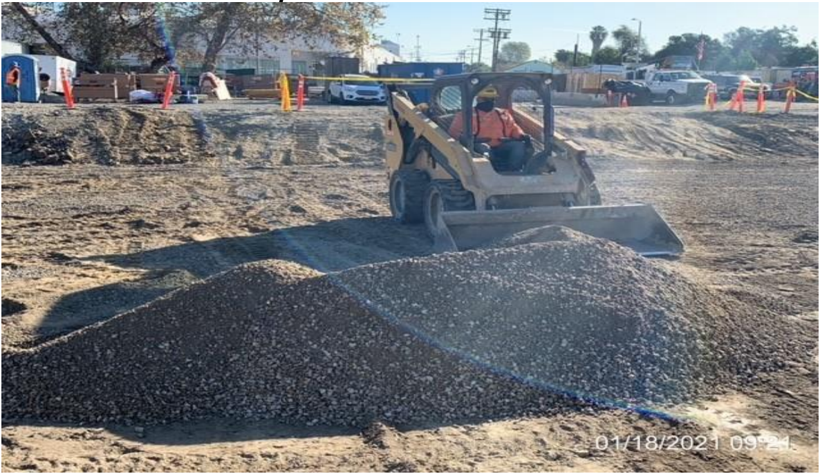
MLK STATION – WSCC placing base and rough grading at park and ride.
