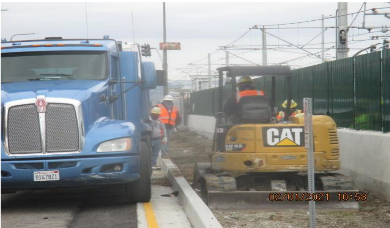
PARK MESA – Continue excavating for swale channel installation along the southbound median curb on Crenshaw Blvd from 59th St to 60th St.
