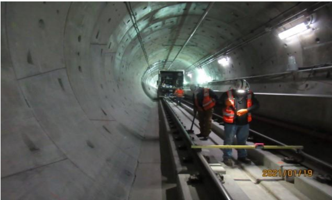
UG4 – HCC in UG4 NB track re-verifying cross level issue for open issues log 000340 after re-adjusting cross level between STA 431+72 & 432+00 (looking south) rework
