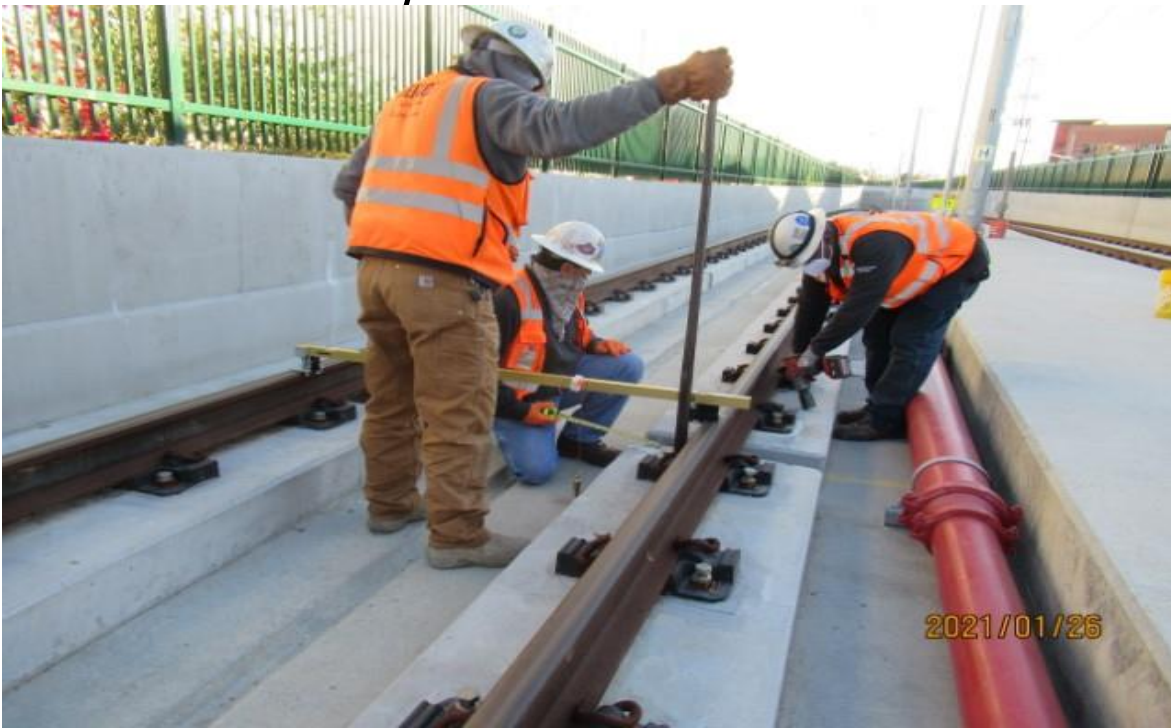
UG3 – HCC adjusting track alignment on survey scribe nail off sets SB track UG3 south portal (looking north) Rework
