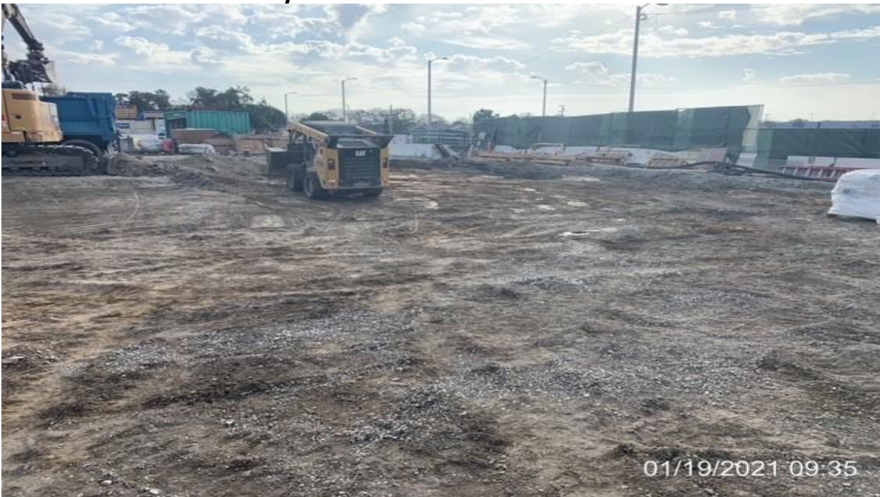
EXPO STATION - Continue excavating/grading and removing existing concrete throughout the entire Park & Ride lot area.
