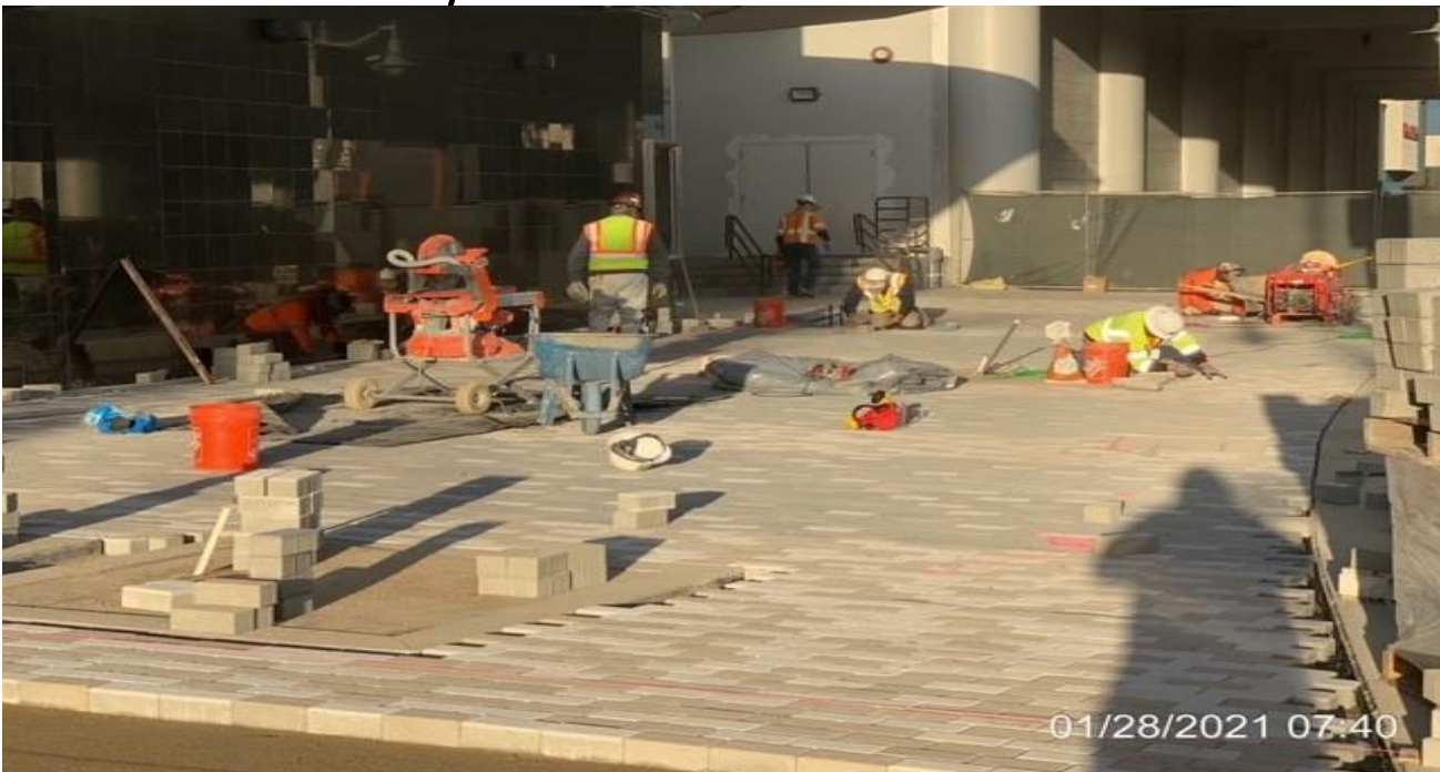
MLK STATION – Continue laying bedding sand and installing brick pavers at the far northwest plaza area.
