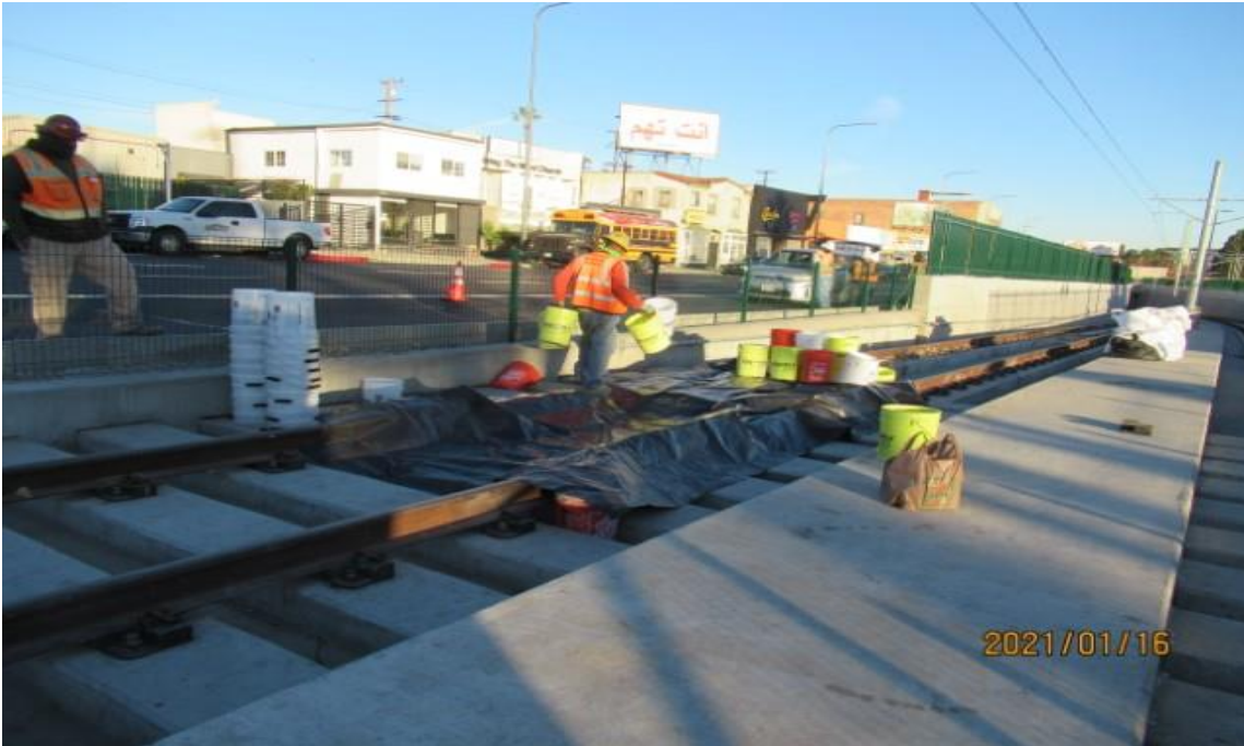
UG3 – WSCC at 48th Street preparing for concrete placement for plinth repair work on SB track (looking northwest) for BIM 360 issues log number 000294 rework
