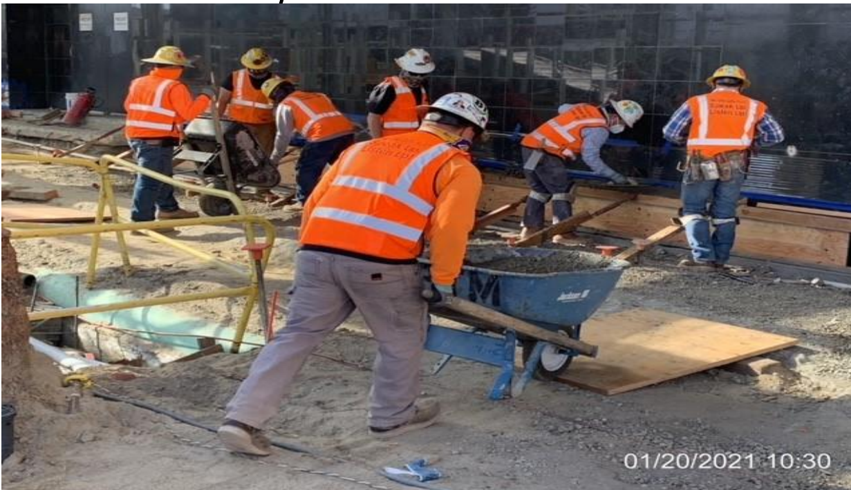
MLK STATION – Placing concrete for the short curb wall along the east side of the Mall at the plaza.
