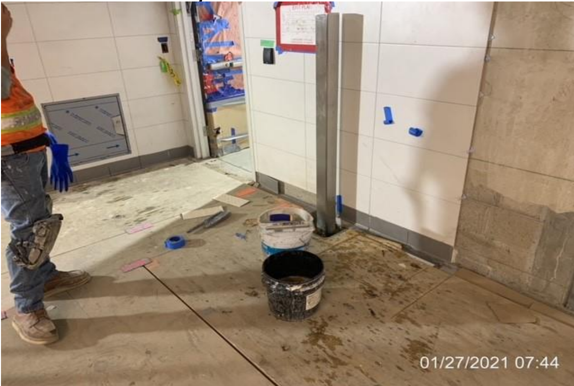
MLK STATION – Premier Tile & Marble installing missing wall tiles and base cover
