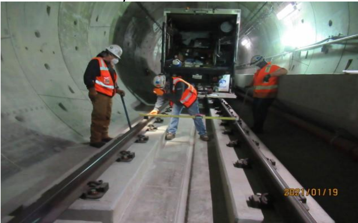
UG4 – HCC in UG4 NB track working on open issues log 000340 cross level out of tolerance between STA 431+72 & 432+00 (looking south) rework
