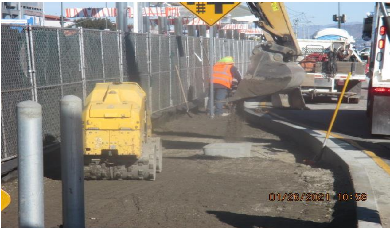
PARK MESA – Placing mortar in preparation for cobble installation along the north and southbound median curbs.
