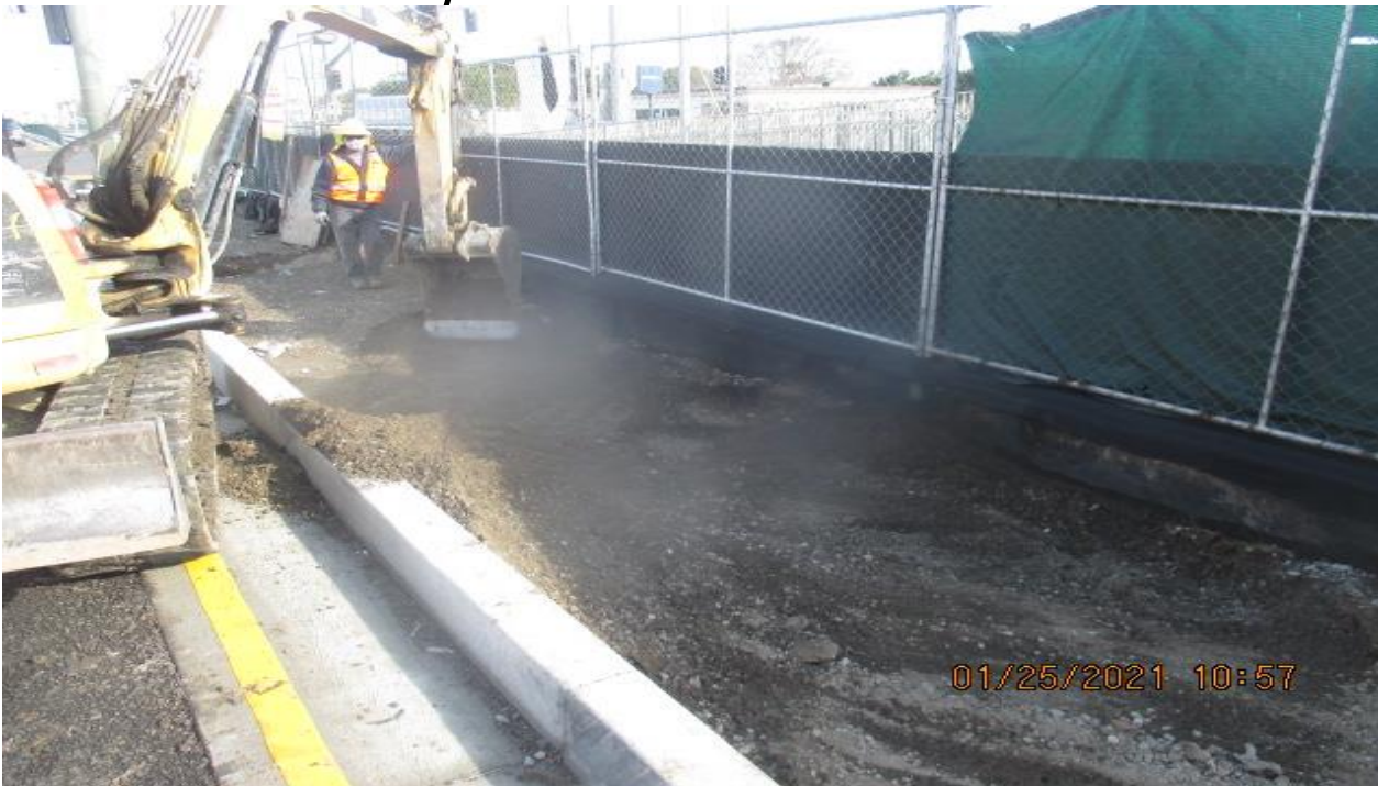
PARK MESA – Excavating for swale channel installation along the southbound median curb on Crenshaw Blvd from Slauson Ave to 59th St.
