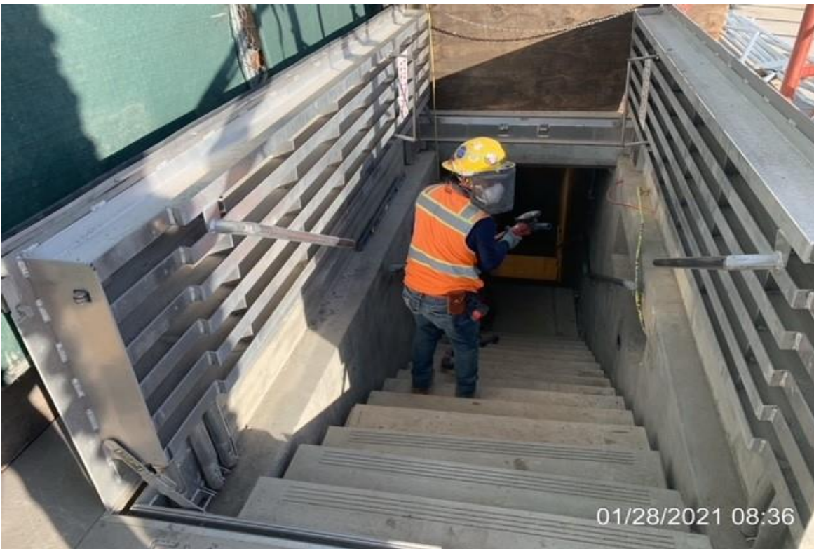
MLK STATION – WSCC finisher grinding and patching surface on ledge for exit hatch #3.
