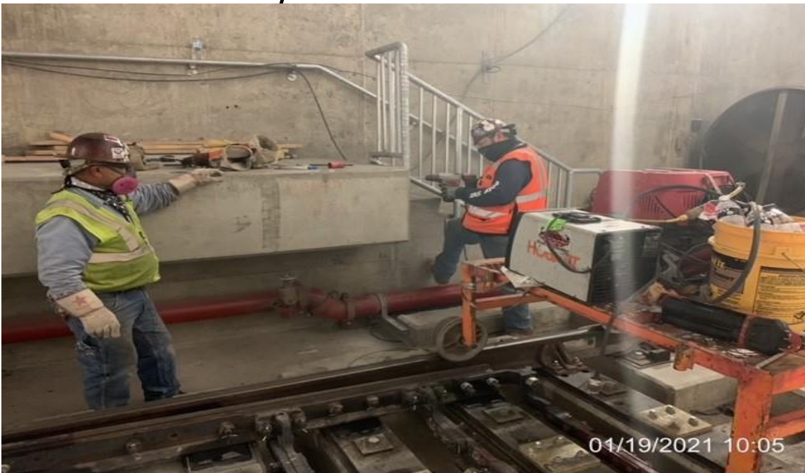
MLK STATION – McMahon installing emergency exit stair guard rail at south portal SB track.
