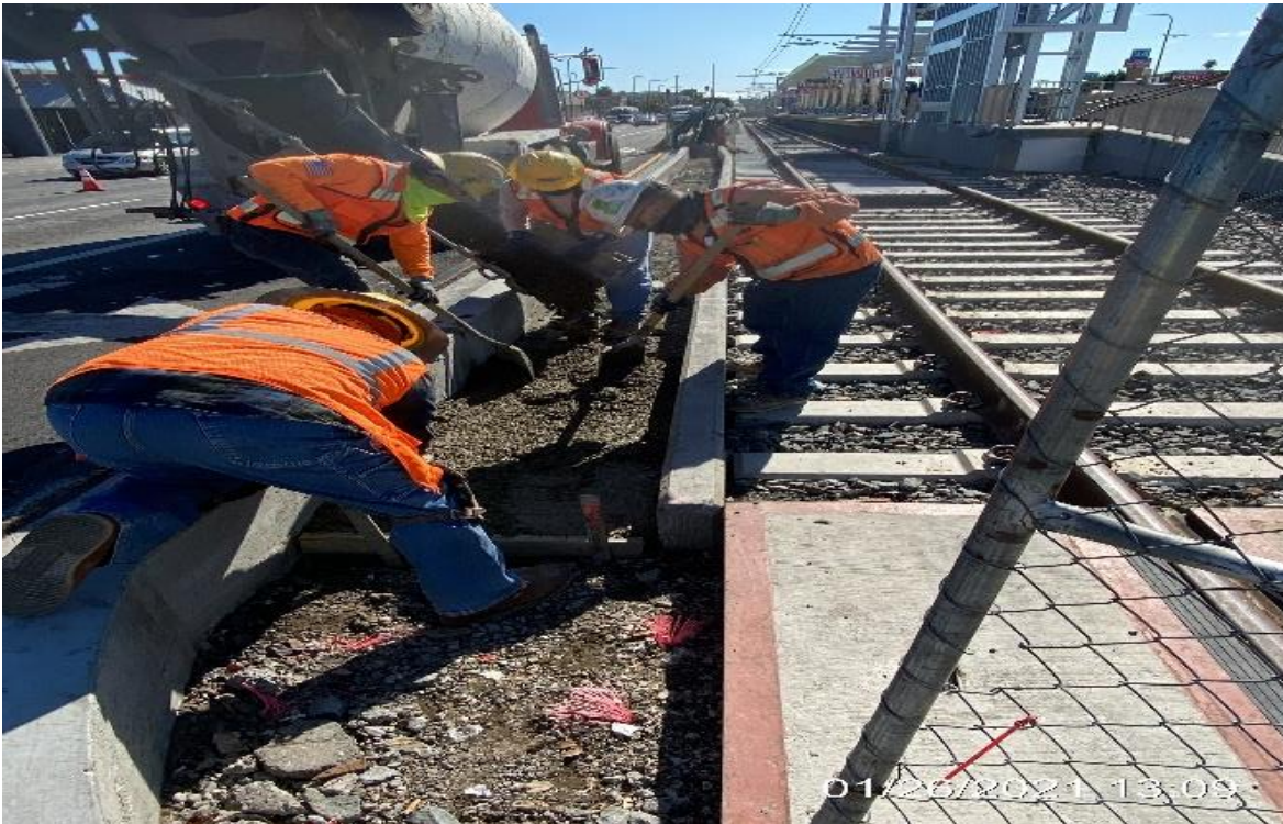
PARK MESA – Placing slurry along the northbound ballast wall near the north entrance ramp.
