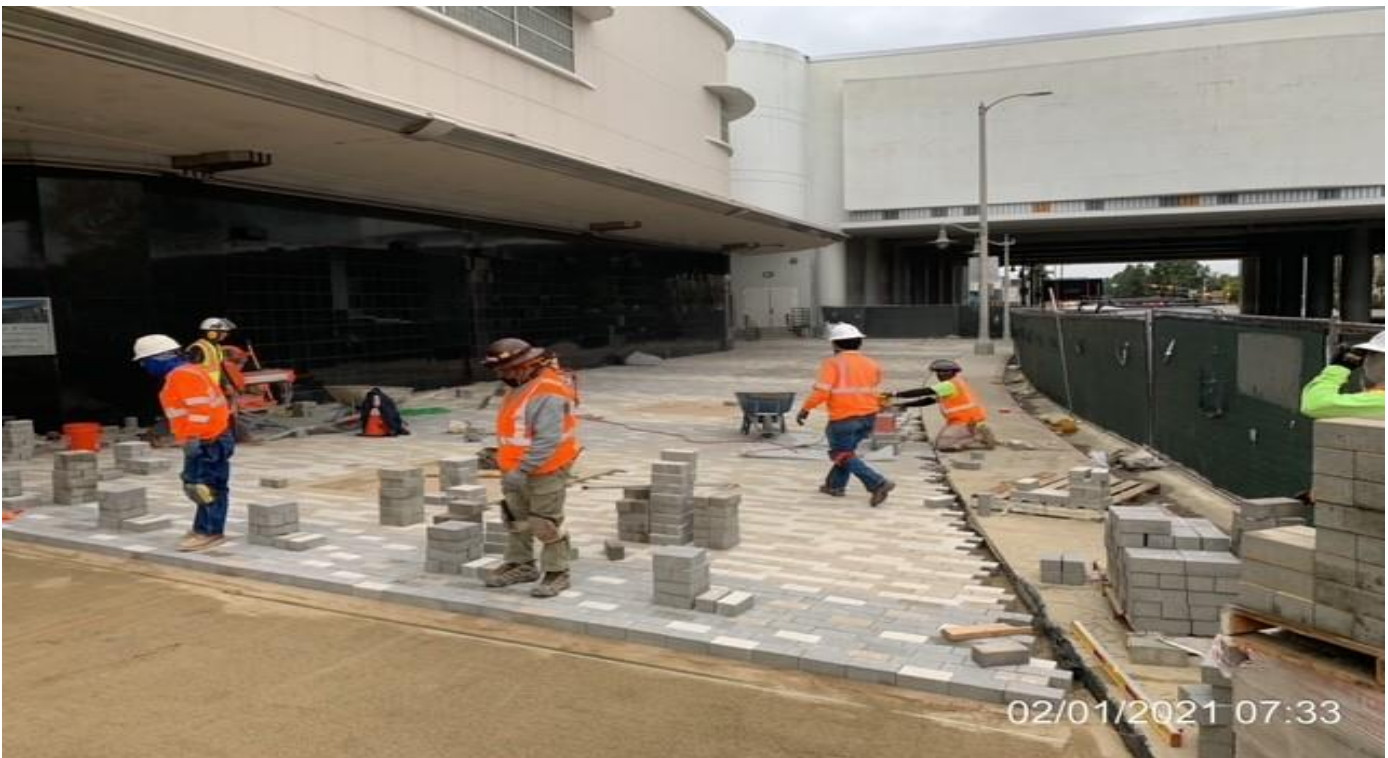
MLK STATION – Continue laying bedding sand and installing brick pavers at the far northwest plaza area.
