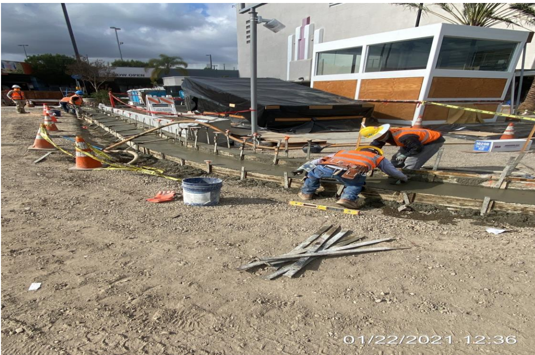
MLK STATION – Placing concrete for new curb and gutter installation along the access road south of the plaza.
