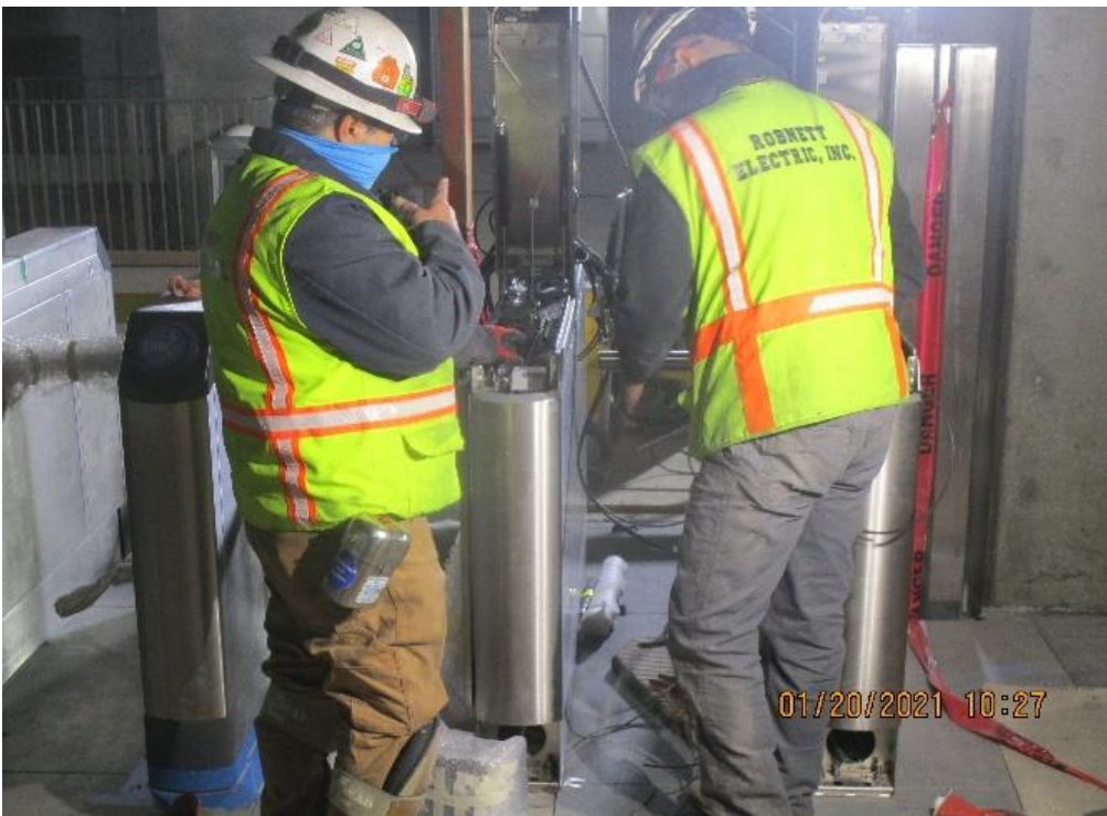
MLK STATION – Continue performing electrical work to the fare gate turnstiles at the Paid & Free Area.
