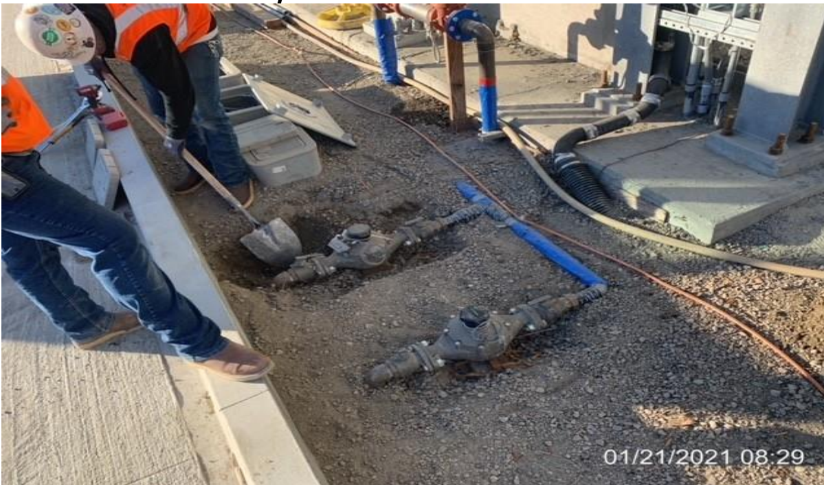
MLK STATION – WSCC crew hand digging to expose (2) water valves for height adjustment
