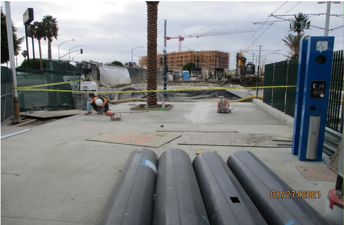
La Brea Station - Cutting expansion joints at the La Brea Station hardscape.
