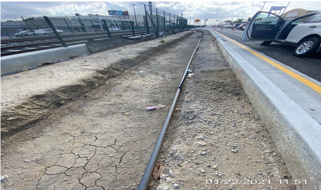
PARK MESA – Placing irrigation along the southbound median of Crenshaw Blvd between 54th St. and 52nd St.
