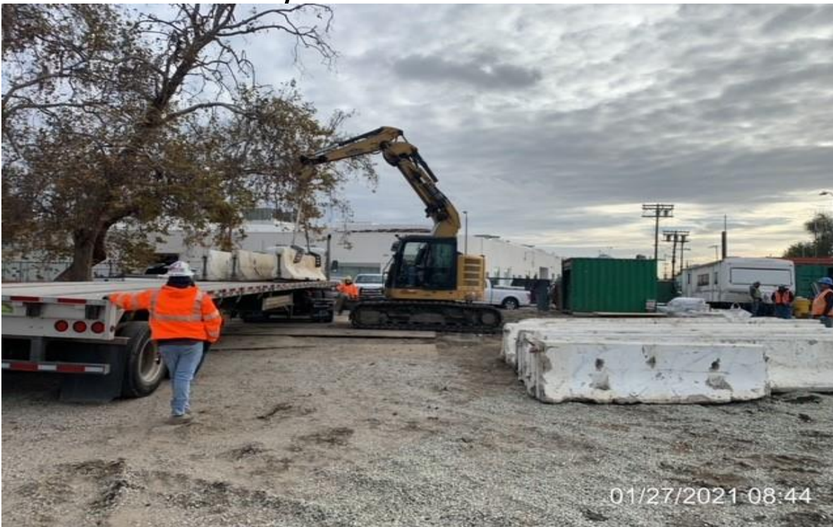
MLK STATION – WSCC crew removing K rail from park and ride yard.
