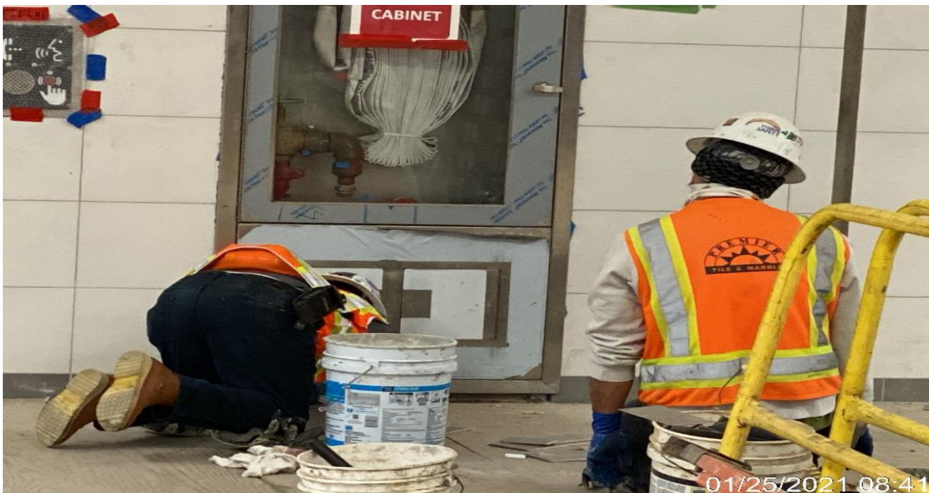
LEIMERT PARK STATION – Installing remaining tile at base cove locations on the platform.
