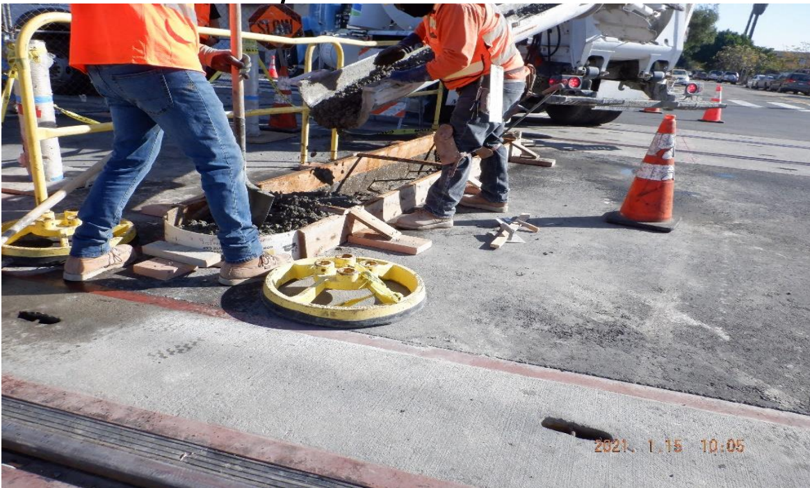
UG3 – STA 317+50 TK#3/SB looking east – pour PCC for raised curb for bollard delineators on Crenshaw Blvd crosswalk with 59th St.
