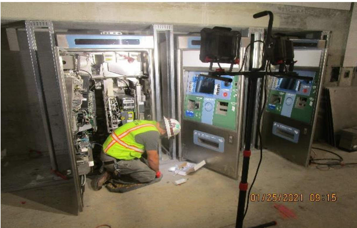
MLK STATION – Anchoring and installing ticket vending machines at the Free Area.
