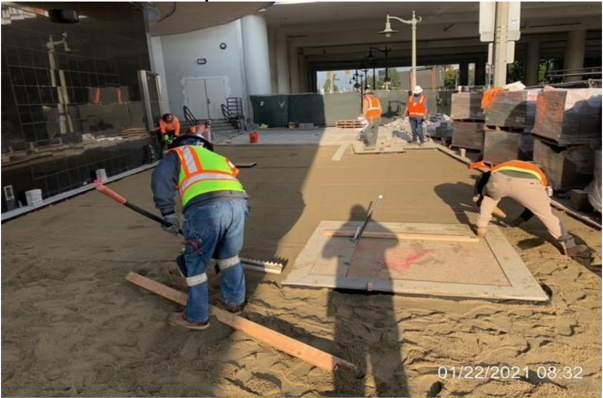
MLK STATION – WSCC crew placing concrete for entrance cove and ADA ramp
