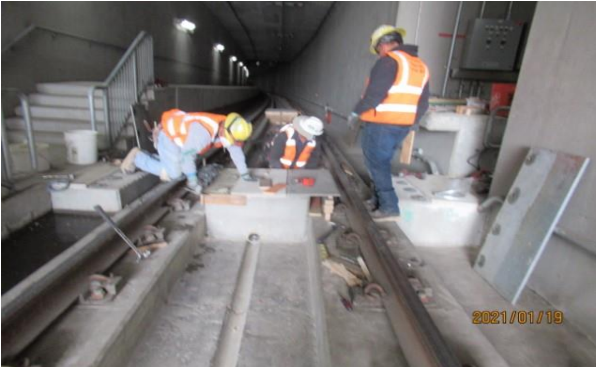
UG4 – WSCC in UG4 NB track STA 371+25 emergency walkway foundations, multiple tasks taking place (looking north) rework
