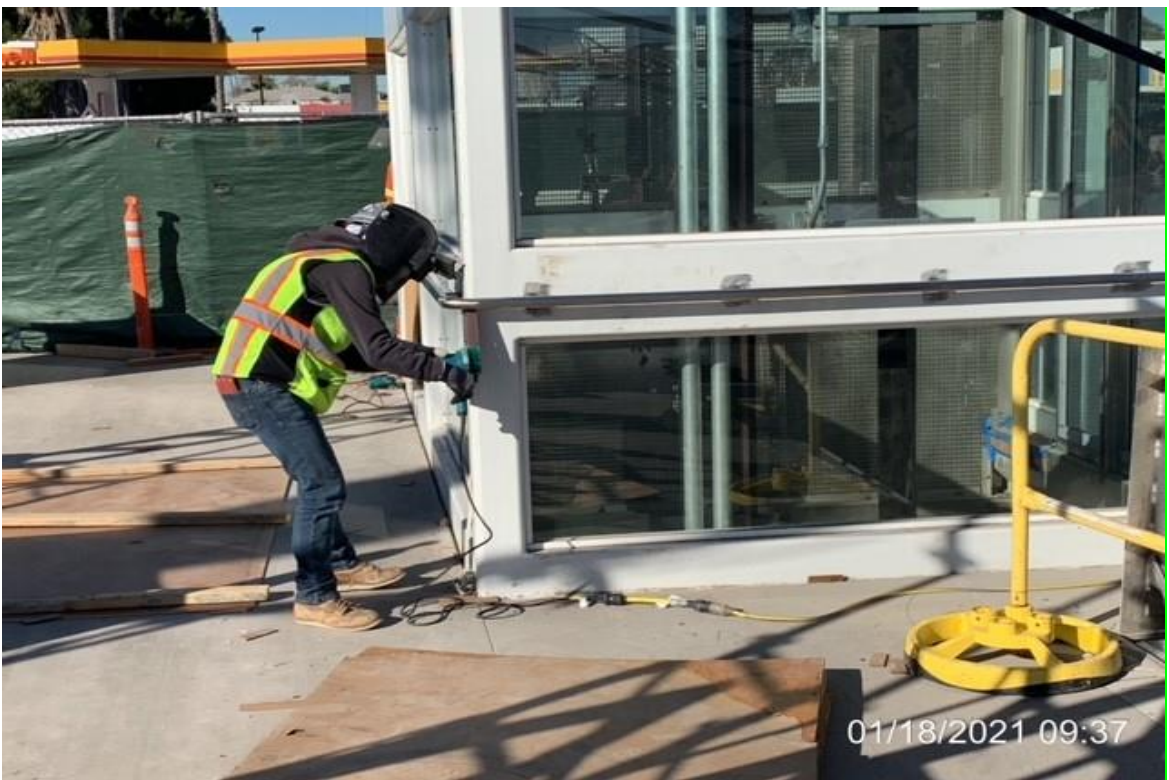
MLK STATION – McMahon grinding to finish stainless steel hand rail for elevator structure #1 and #2.
