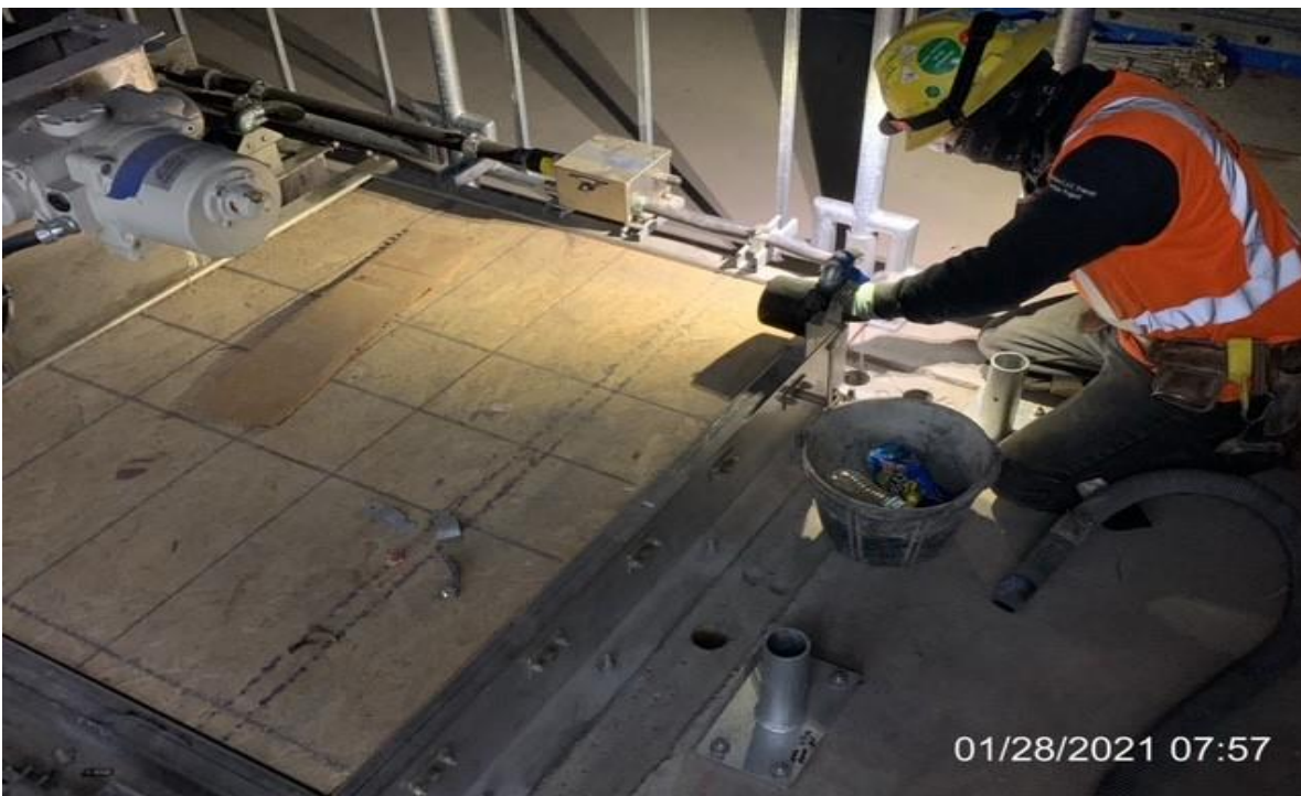
MLK STATION – WSCC finisher filling and patching holes not used for guardrail at north EVF room
