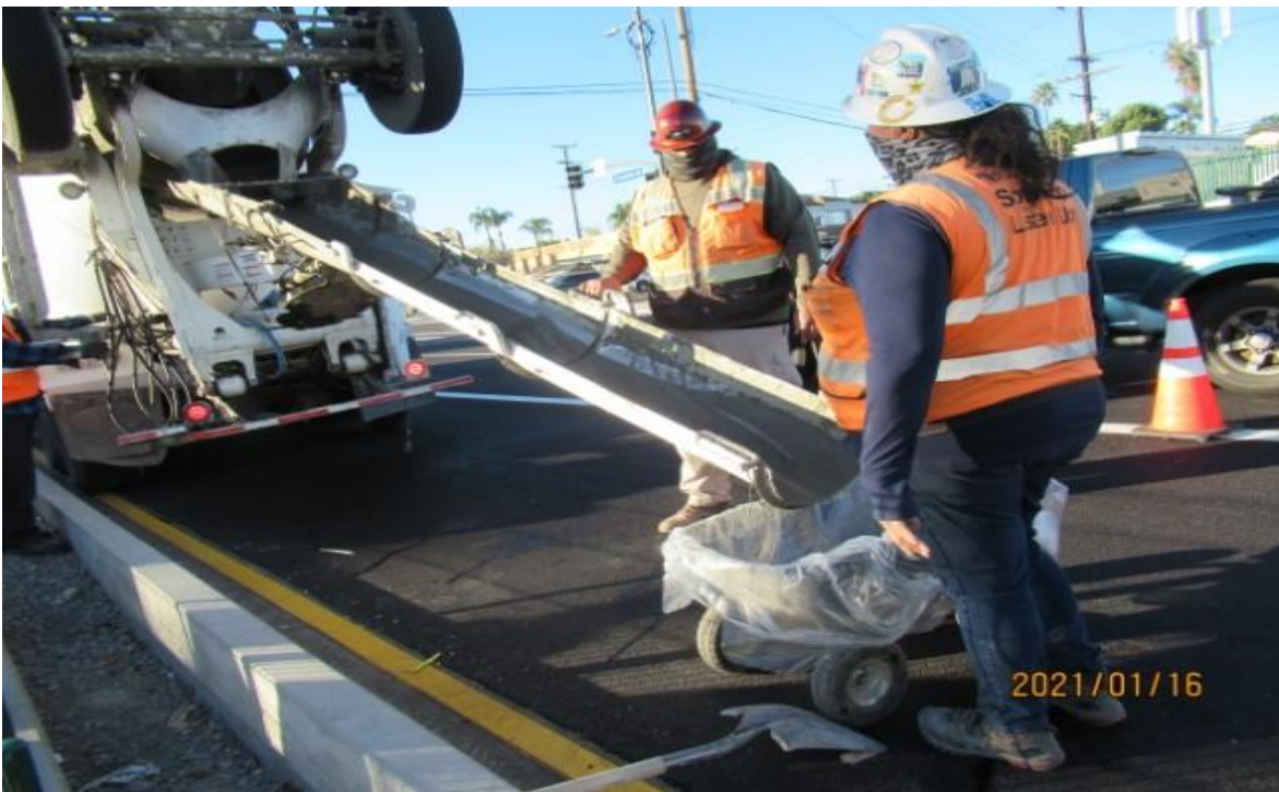
UG3 – RMA Concrete Inspector, collecting concrete samples for break test cylinders at 48th Street (looking southwest) for BIM 360 issues log number 000294 rework
