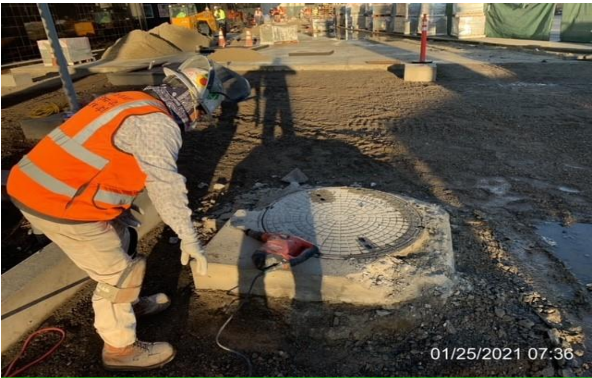
MLK STATION – WSCC finisher chipping out damaged manhole encasement
