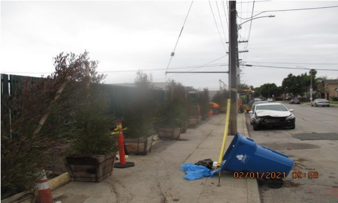
PARK MESA – Installed trees and shrubs along the Victoria Auxiliary fence on eastbound 67th St and Crenshaw Blvd.
