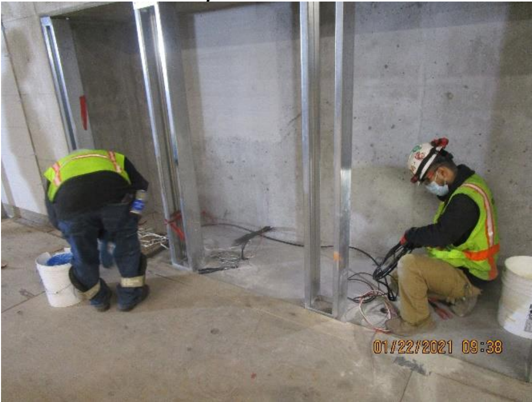
MLK STATION – Preparing for ticket vending machine installation at the Free Area.
