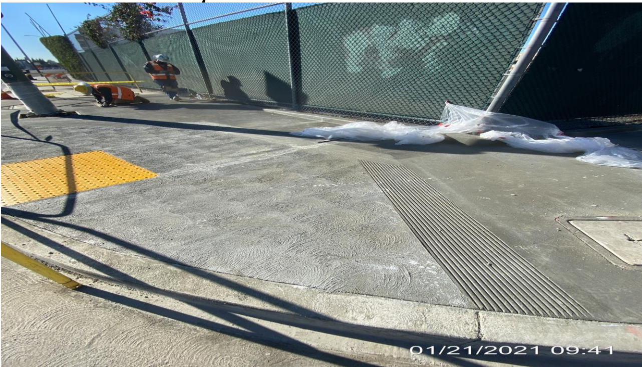
PARK MESA – Saw cutting control joints for new sidewalk and ADA ramp installation on the southwest corner of 60th St and Crenshaw Blvd.
