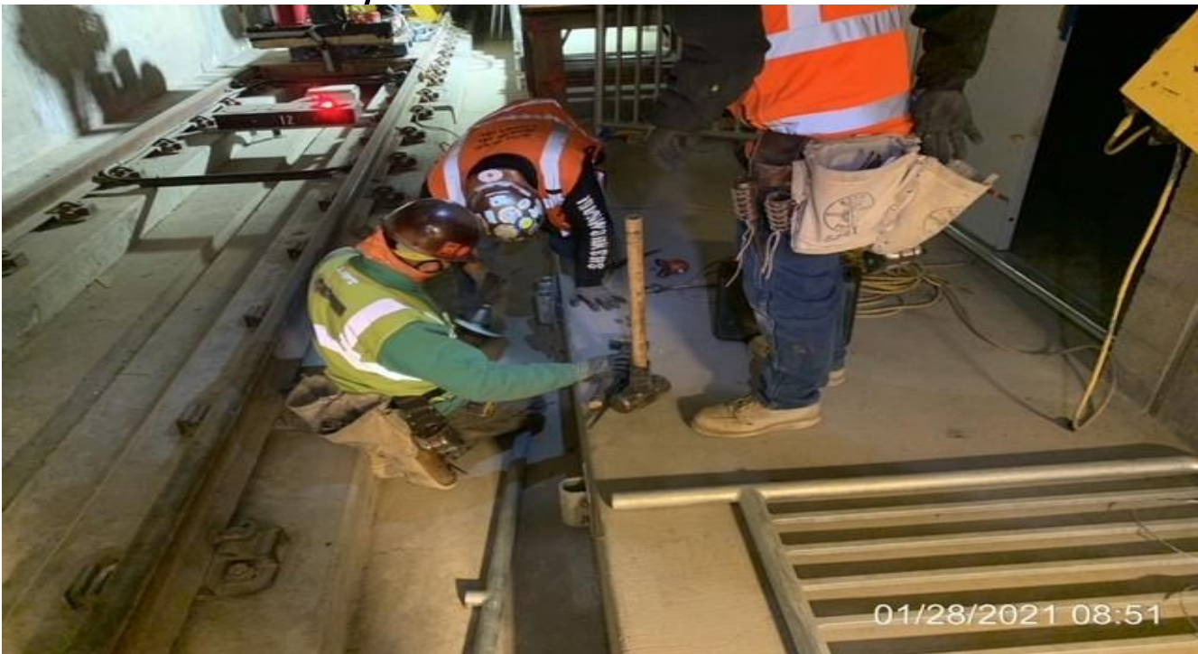
EXPO STATION – Continue installing guardrails along the northbound emergency walkway of the North back of House at the invert level.
