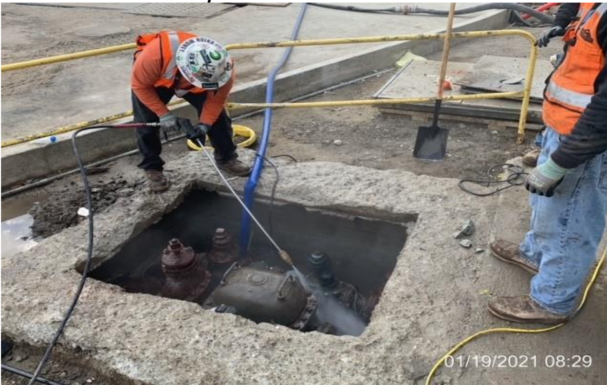
MLK STATION – WSCC crew power washing residual concrete from encased water service lines
