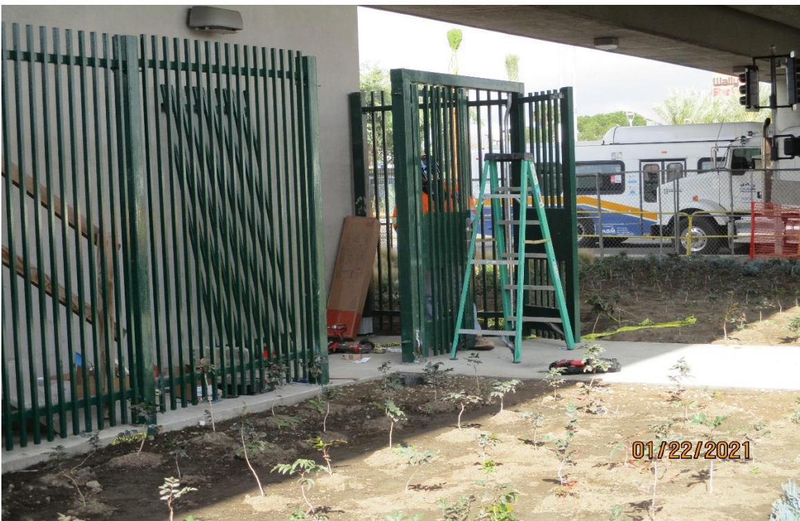
AVIATION/CENTURY- Door hardware installation at the SW corner of Aviation and Imperial.
