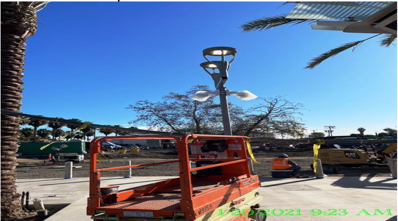
EXPO STATION– Installed domes to all the CCTV cameras mounted on pedestrian light poles throughout the plaza.
