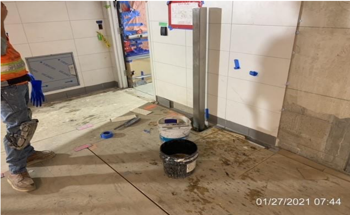
MLK STATION – Installing remaining tile at base cove locations throughout the Free Area.
