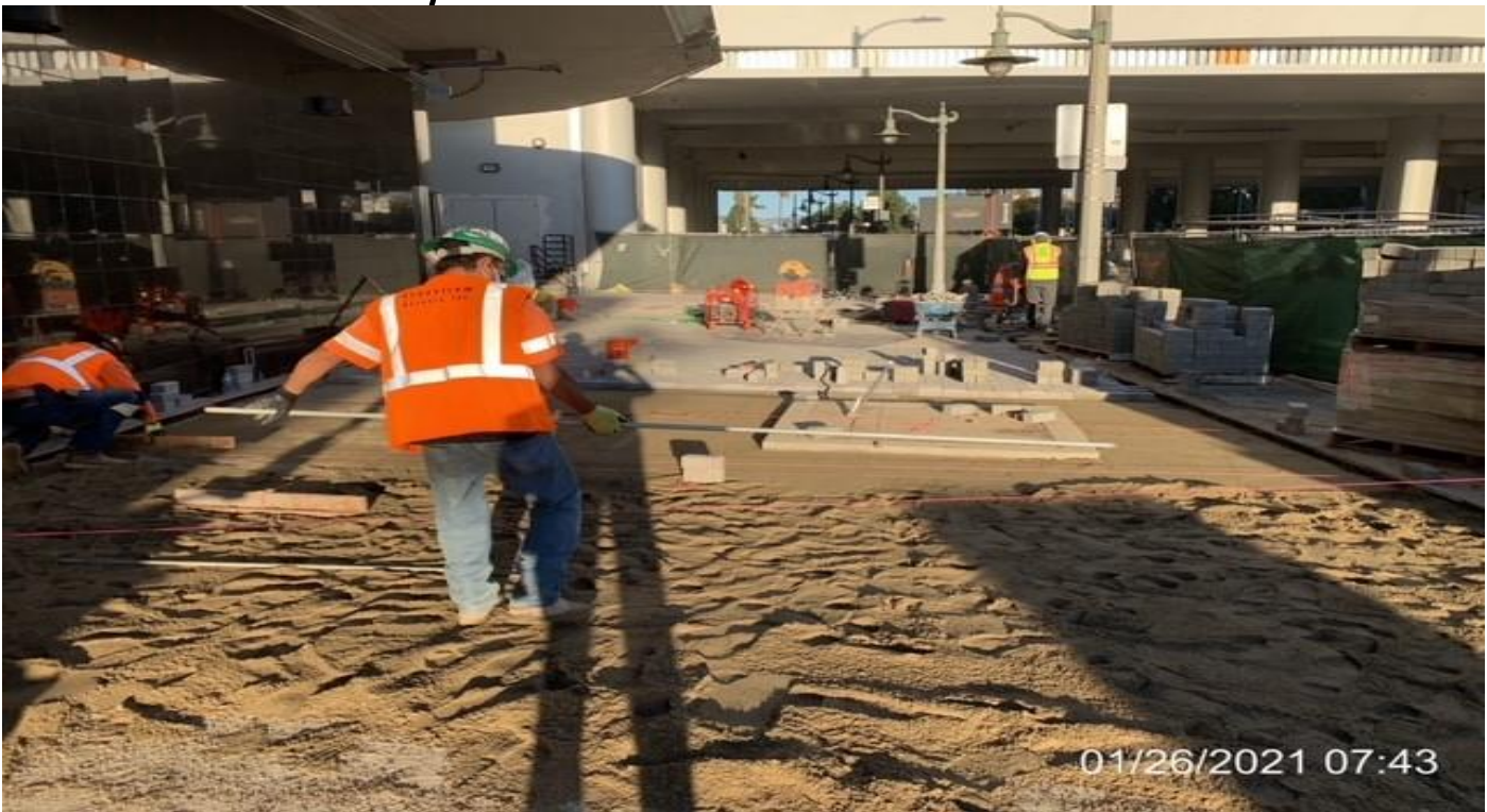
MLK STATION – Continue laying bedding sand and installing brick pavers at the far northwest plaza area.
