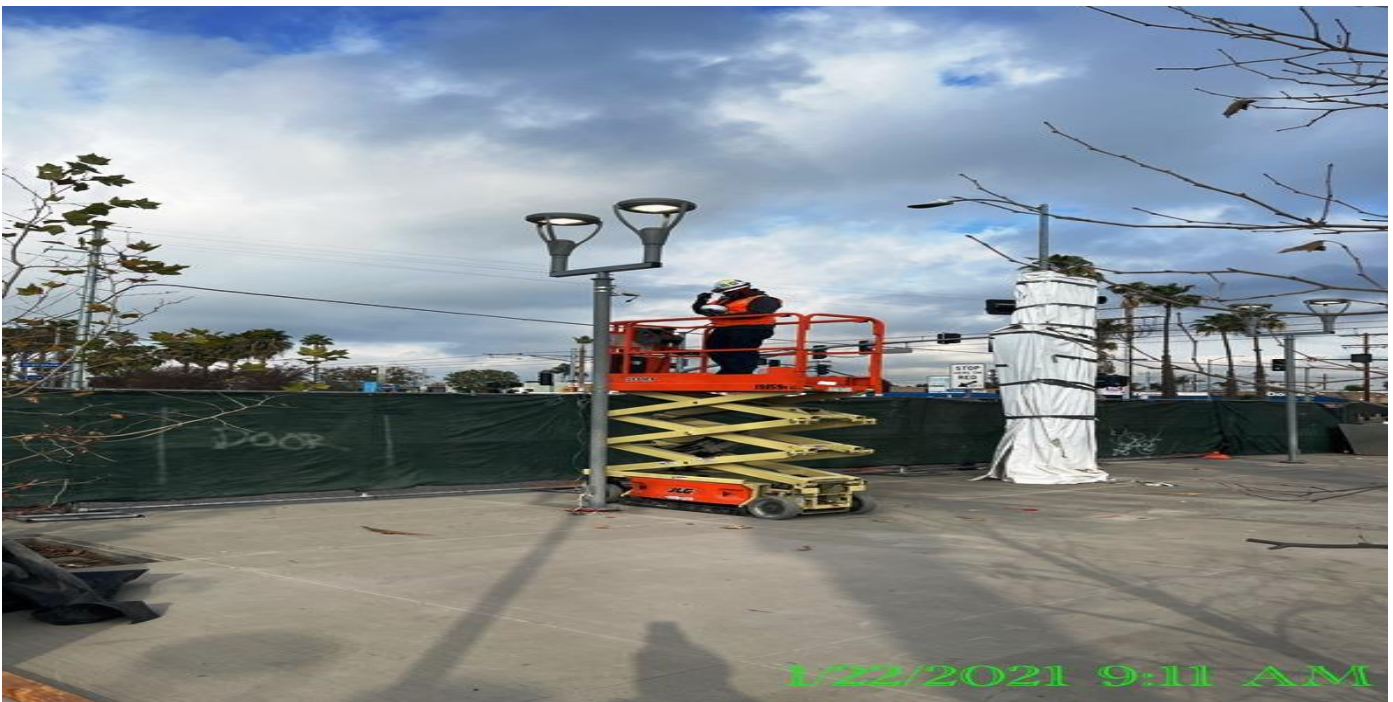
EXPO STATION – Continue dome installation to all the CCTV cameras mounted on pedestrian light poles throughout the plaza.
