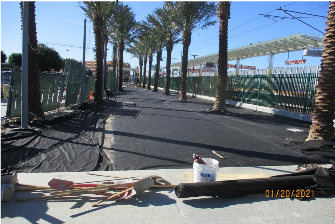
La Brea Station - Weed deterrent fabric placed prior to decomposed granite at the La Brea Station.
