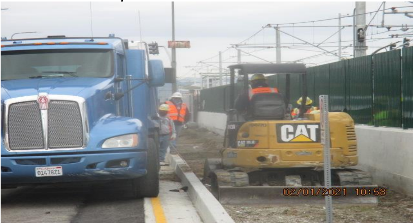
PARK MESA – Continue excavating for swale channel installation along the southbound median curb on Crenshaw Blvd from 59th St to 60th St.
