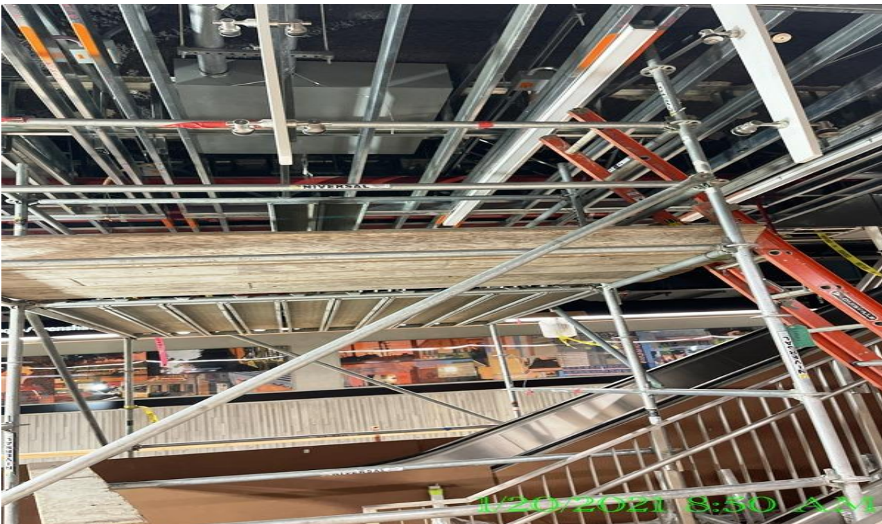
EXPO STATION – Continue LED light fixture installation at the platform ceiling grid.
