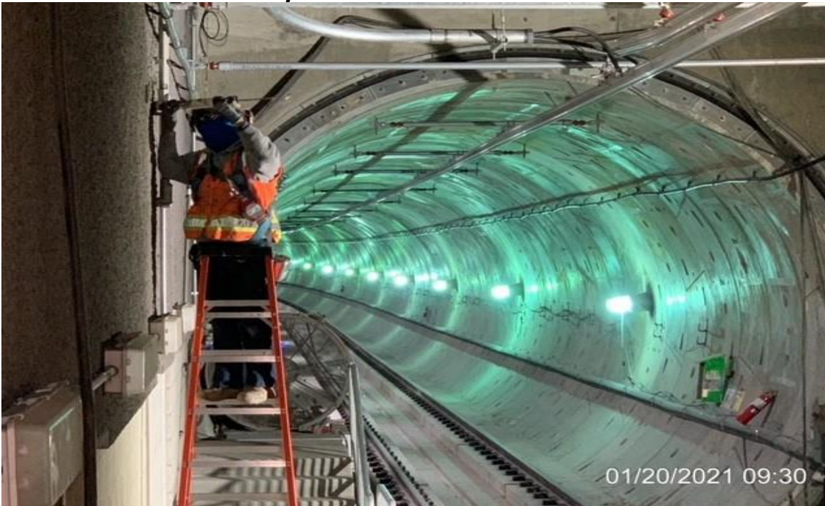
MLK STATION – Bielski fire proof caulking unfinished penetrations at invert level back of house NB side.
