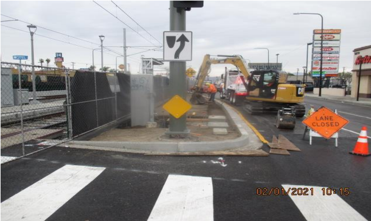
PARK MESA – Excavating in preparation for cobble installation along the northbound median curb.
