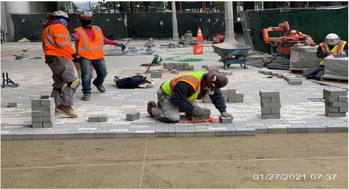
MLK STATION – Continue laying bedding sand and installing brick pavers at the far northwest plaza area.
