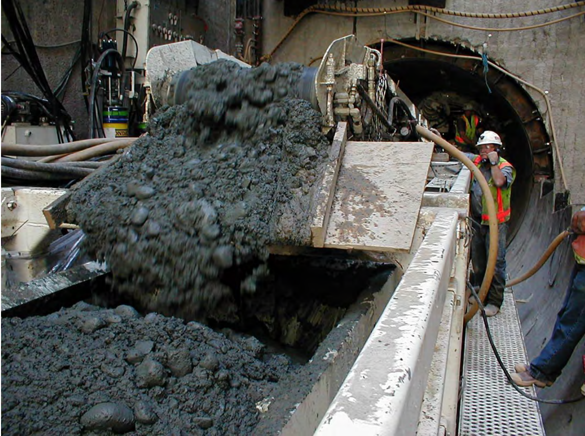
Figure 12-3. Alluvium of the Lakewood Formation, with cobbles, falling off a conveyor during excavation of the ECIS Tunnel.
