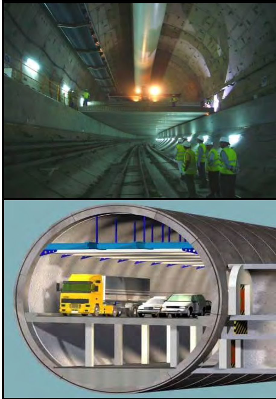
Figure 12-8. Roadway slab construction for the Calle 30 tunnel in Madrid (top) Schematic showing the final use of the tunnel (bottom).
