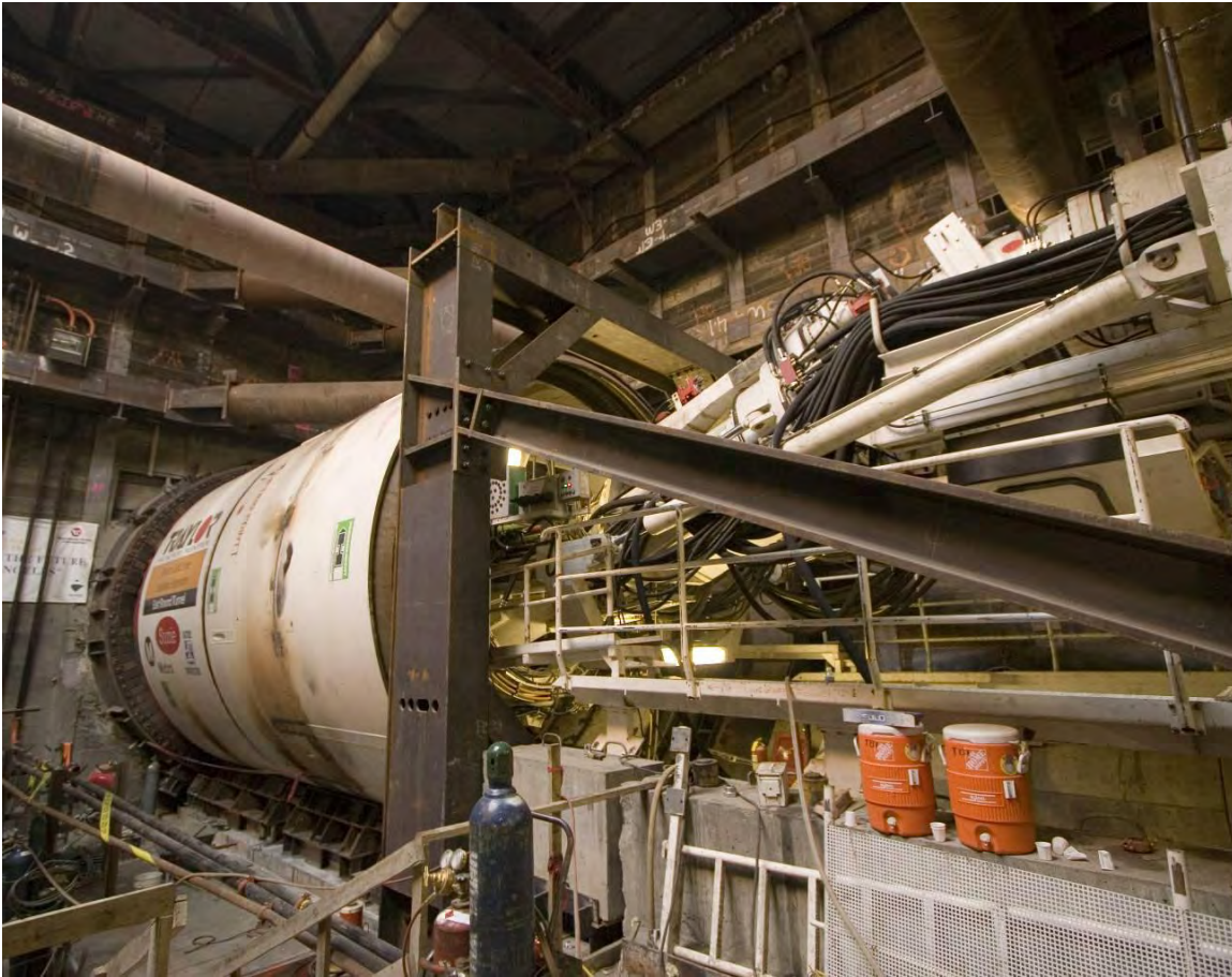
Figure 12-5. TBM Being Launched for the Metro Gold Line Eastside Extension in Los Angeles.
