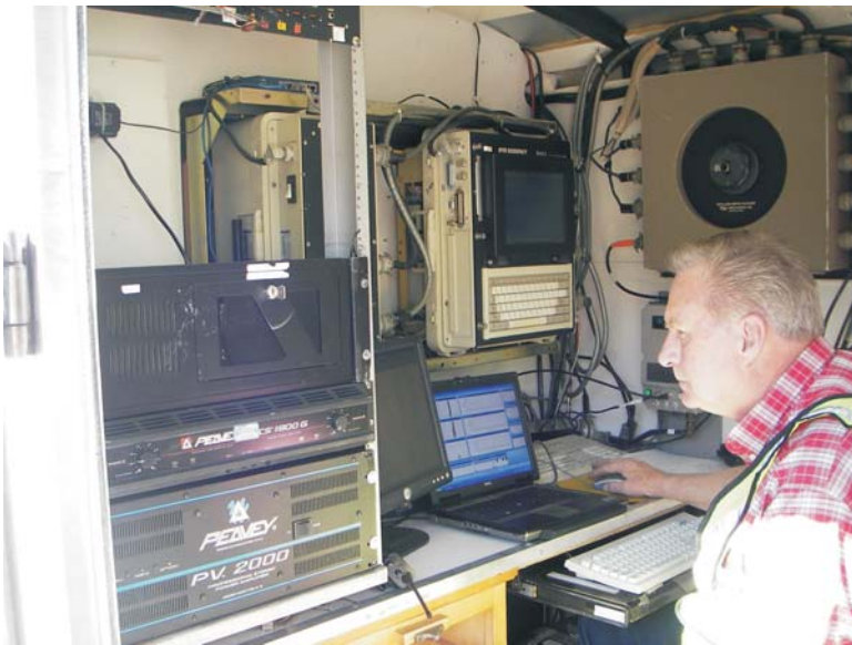
SEISMIC RECORDING SYSTEM
