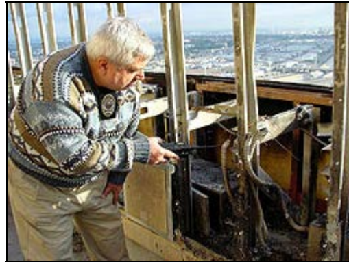
Security Director Dan Cowden inspected the damage shortly after the fire was extinguished.
