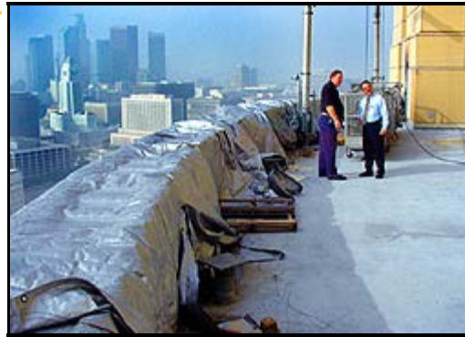
Bob Skarseth and Bob Ketring of General Services take a look at the area where the Gateway building parapet will be repaired.
