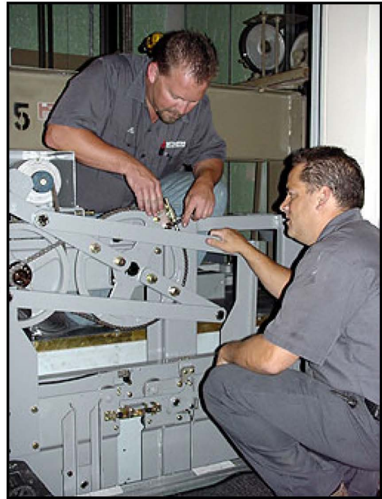
^ Mechanics Mike Mershon and Nick Trujillo of Mitsubishi Electric adjust a new heavy-duty door operator on an elevator in the low-rise bank at MTA Headquarters. Modernization of elevators in the high-rise bank is scheduled to start in July. PHOTO BY BILL HEARD.
