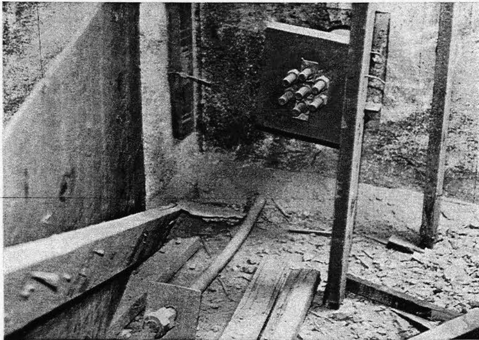
Inside cell opposite of previous pictures, equalizing bolt in fore ground.
