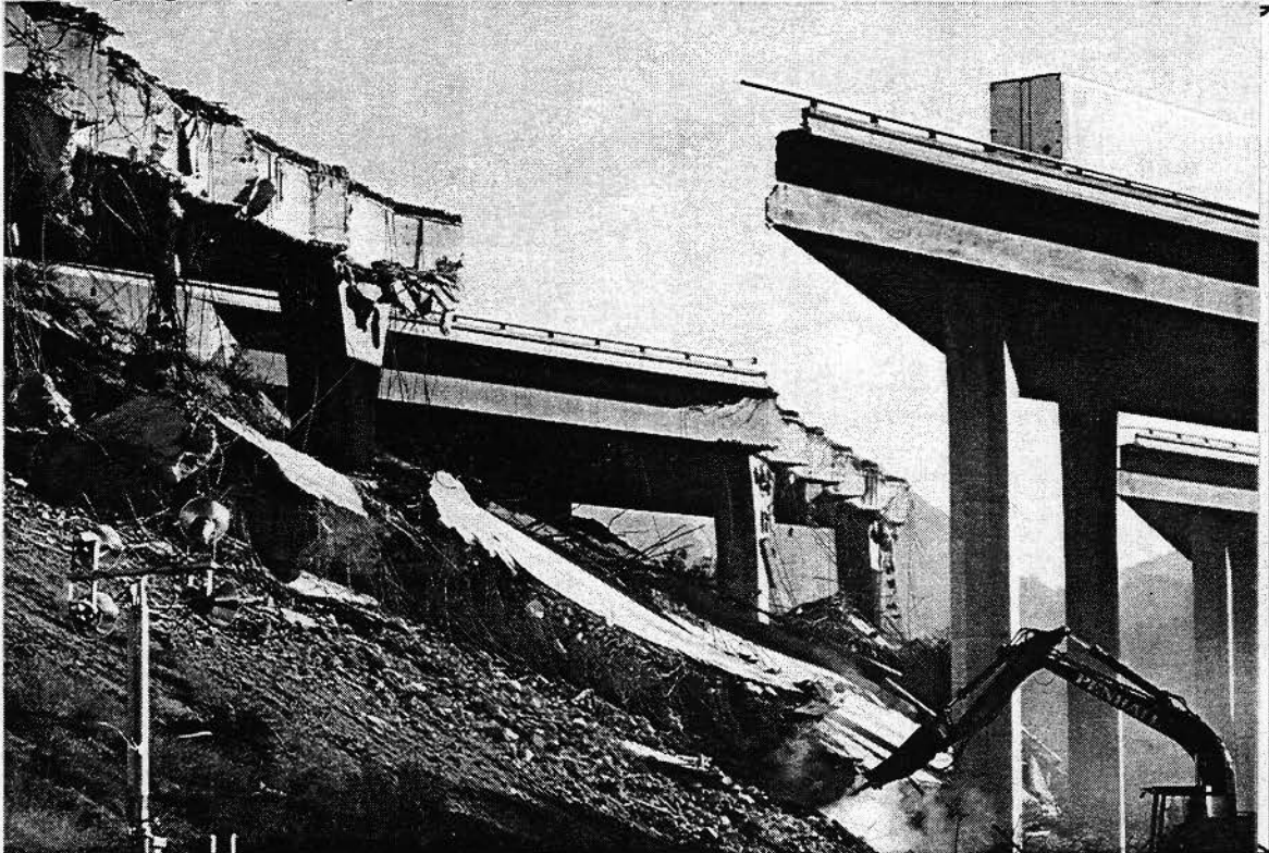
Gavin Canyon Bridge 53-1797R/L 7-LA-5-R47.83 3-2-JSM Demolition in progress, span 4, southbound structure
