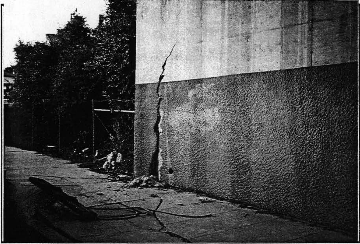
Rinaldi Street Undercrossing Crack in North Bin Wall.
