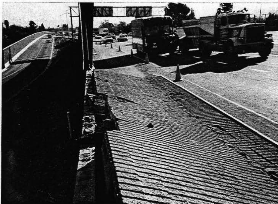
Collapsed Soundwall on WB Route 101 near Interstate 405
