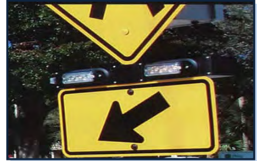
Rectangular Rapid Flashing Beacons are installed between the crossing sign and the supplemental arrow. Source: FHWA.
