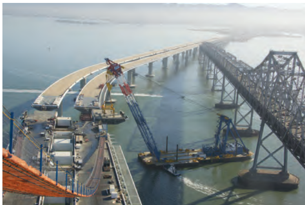
Lifting of a segment of the new Bay Bridge as seen from the new Bay Bridge tower.
