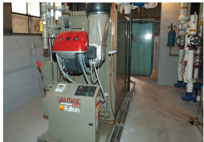
Vantage Hydronic boiler for the District 9 office.
