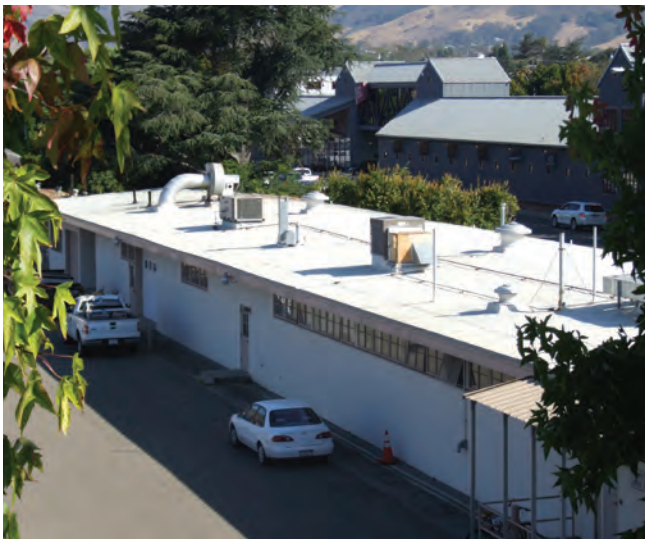
A view of the cool roof on a District 5 building in San Luis Obispo.
