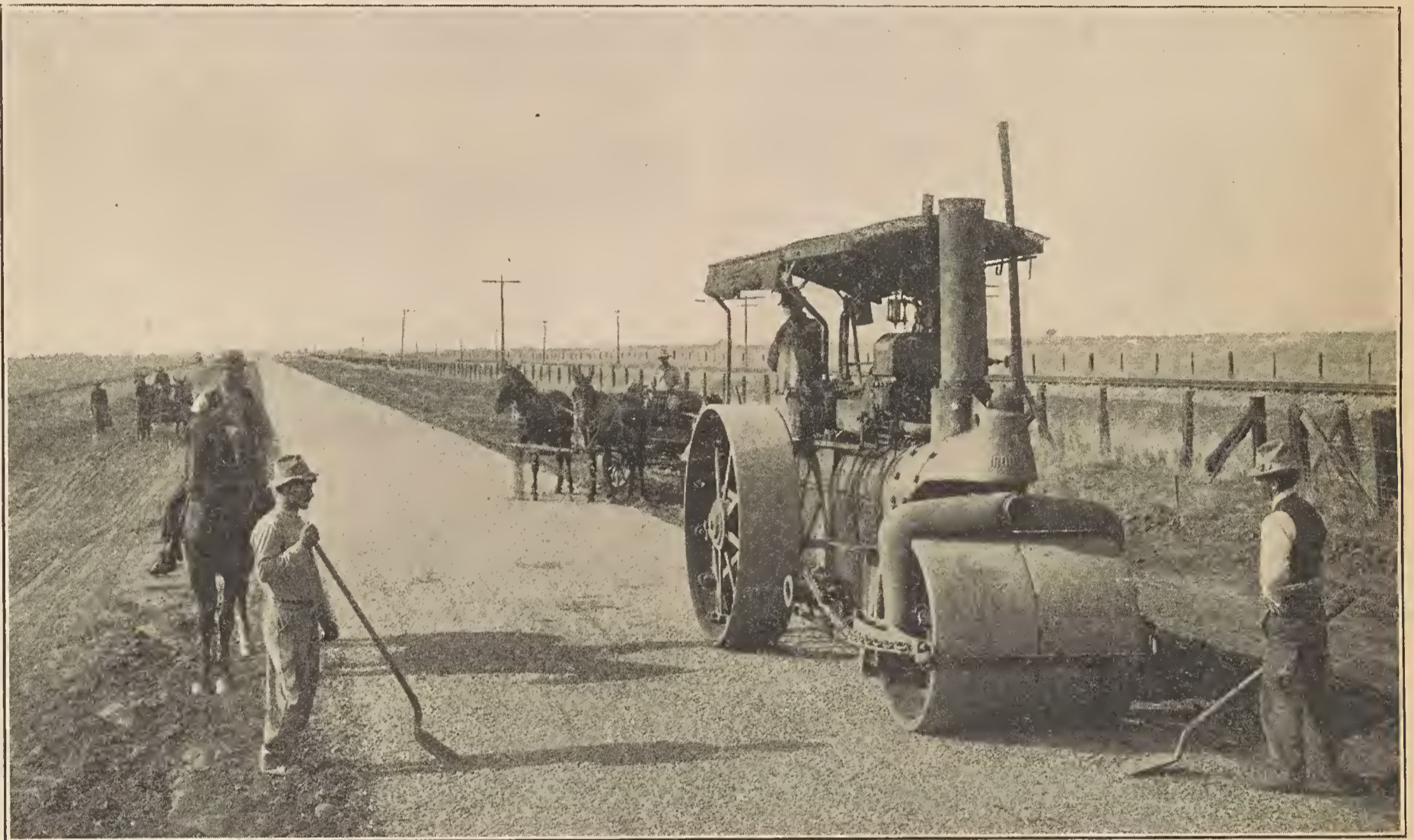
Three Miles of California State Highway Near Marysville, Yuba County, Ready for Surfacing.
