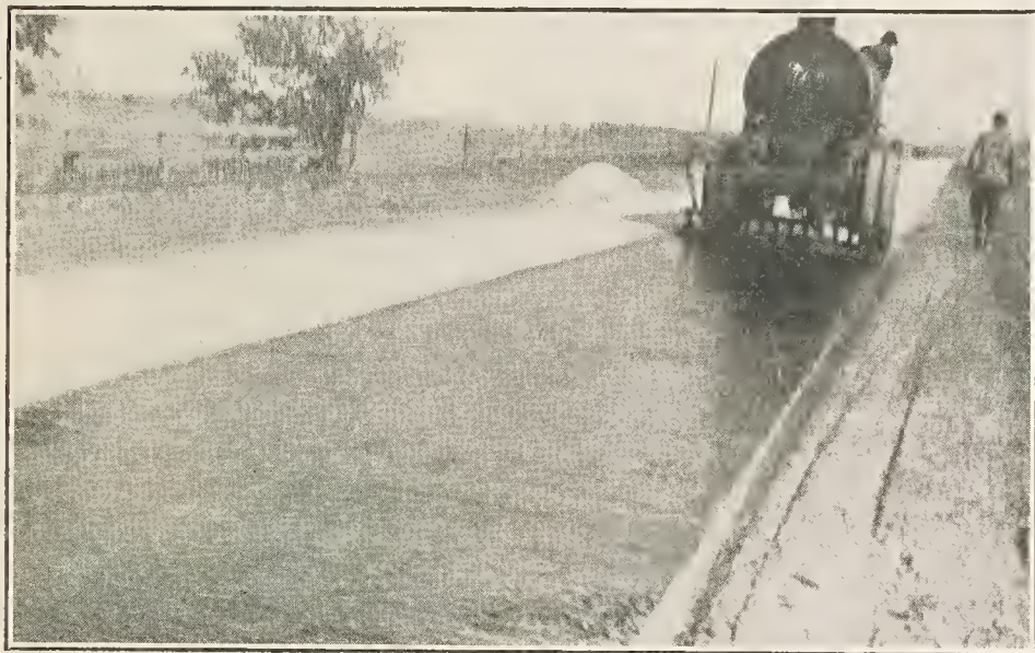
Motor Oil Spraying, State Highway, Los Angeles County.
