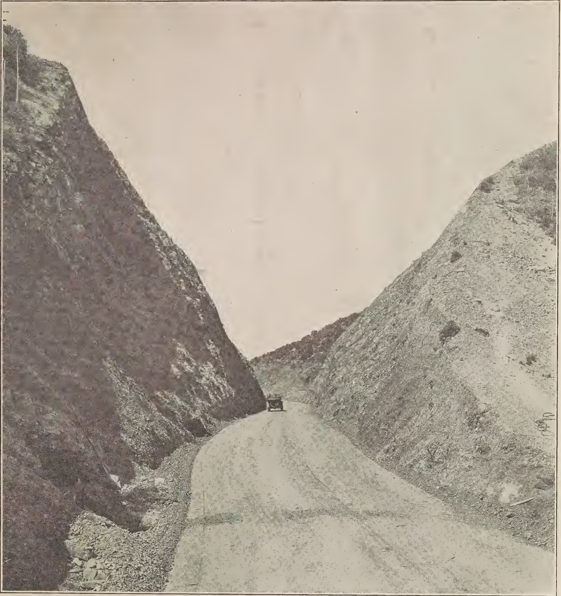
One of the many heavy cuts on the Castaic Ridge Route between Bakersfield and Los Angeles, depth 110 feet. Over one million cubic yards of excavation were necessary in the construction of two sections of this road.
