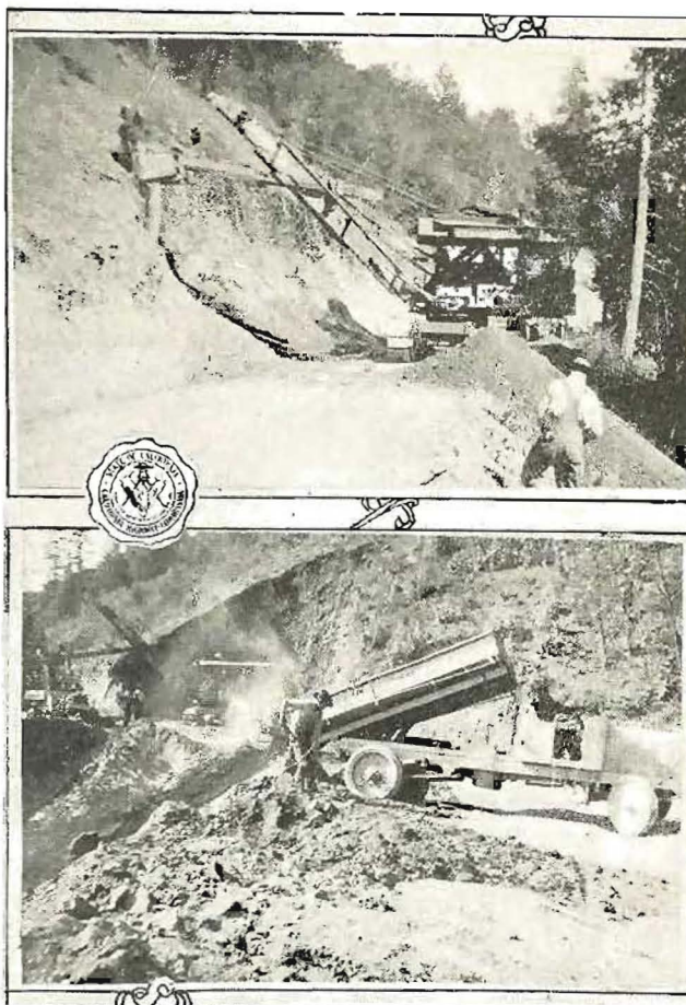
MAKING THE REDWOOD HIGHWAY SAFE—Steam shovel and truck outfit busy in Division 1 widening the Redwood Highway, Mendocino County, a federal aid route.
