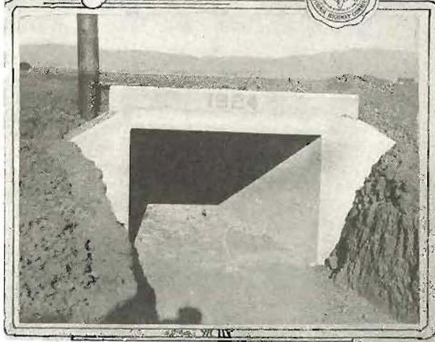
IMPROVING DRAINAGE—Large culvert constructed near Irvine, Orange County, to assist the completion of a cross-county drainage system. The upper view shows traffic using the highway unhampered by the construction under way.
