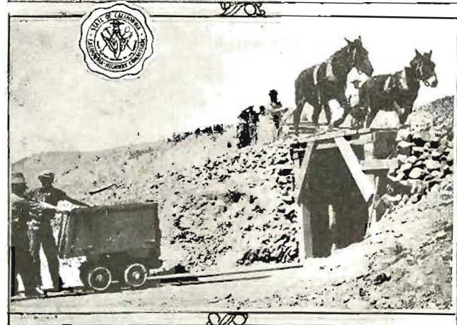
DIVISION IX BUSY—Rock crushing plant of Division Engineer F. G. Somner getting out surfacing material for a section of the state highway in the Sherwin Hill district, Mono County.
