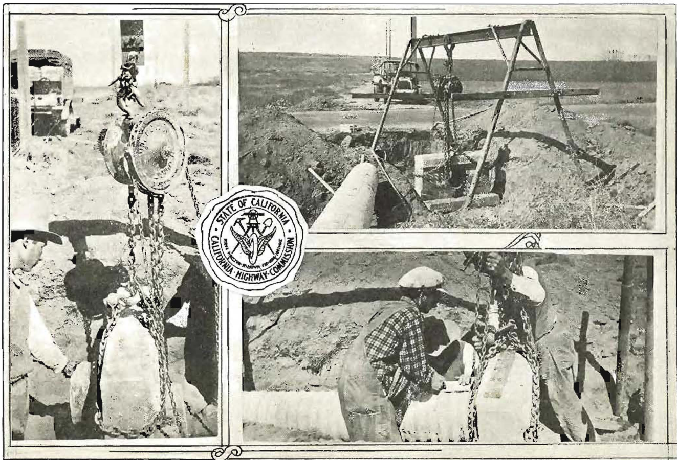
ECONOMICAL CULVERT EXTENSION, DIVISION VII.—Upper right, hoisting frame, carrying a trolley with two-ton chain hoist, built at the Lankershim shops for moving concrete headwalls during culvert extension operations. Other views show the process of moving out the headwall and clamping of the pipe extension in place.
