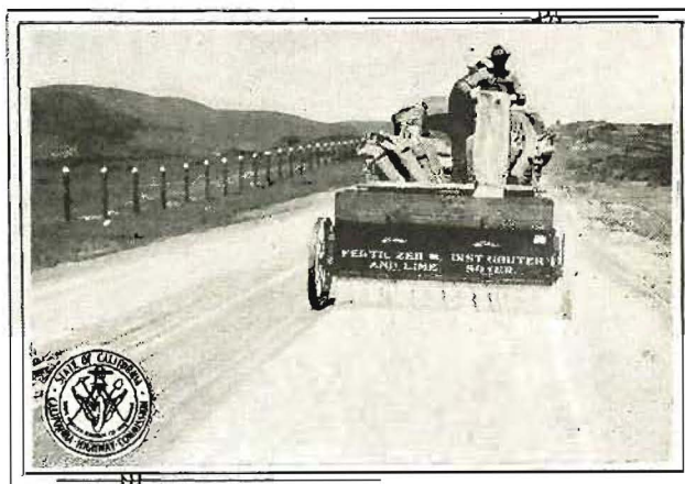
SPREADING CALCIUM CHLORIDE—Methods used in Division IV to spread calcium chloride on the Skyline boulevard, south of San Francisco. This chemical absorbs moisture from the air, binding the surface of the road and lessening the dust.
