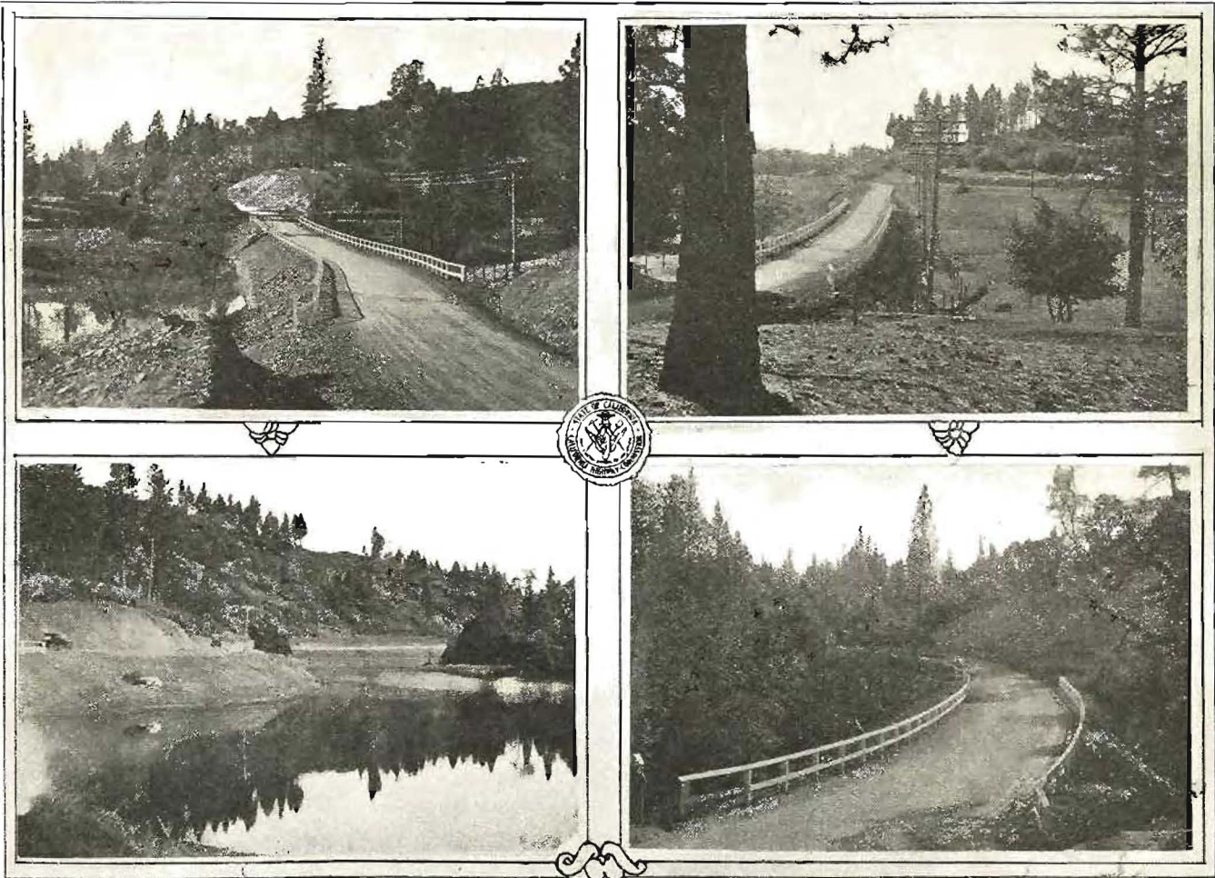
Construction on the Victory highway: Scenes on the recently completed unit of the state highway between Auburn and Colfax, in Division III. The views show the improved alignment, width, and high standards of the new construction.
