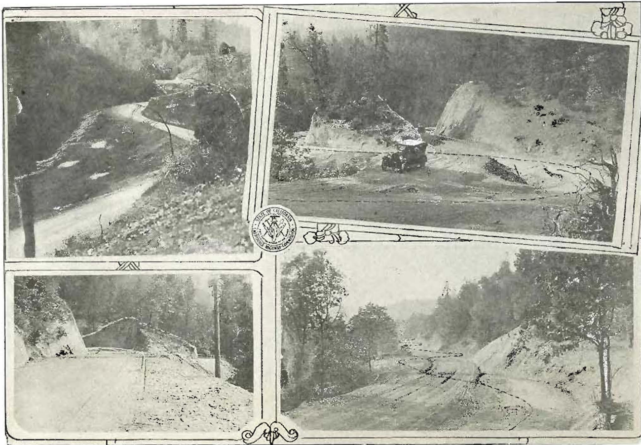
STRAIGHTENING THE PACIFIC HIGHWAY—Upper left, old grade cleared for new work; upper right, cut and fill eliminating sharp curve, dotted line being center line of former grade; lower left, grade and line change, old grade at right; lower right, elimination of curves by cuts and fills, dotted line showing former location.
