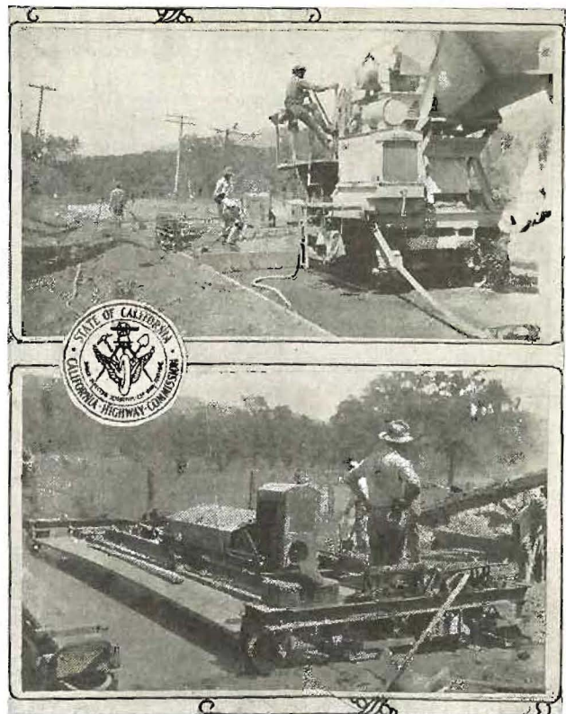
PAVING IN THE "VALLEY OF THE MOON"—Views of paving operations between Beltane and Schellville, Sonoma County. Mechanical spreader and tamper in operation, insuring a smooth surface for the pavement. (Photos by Division IV.)
