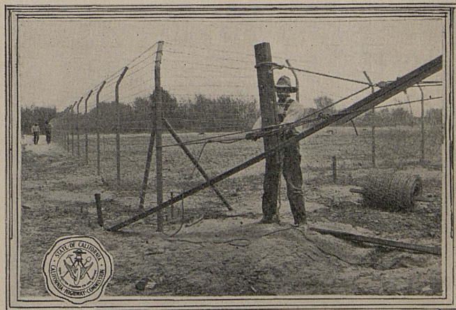
DISCARDED PIPE NOW FENCE POSTS—Division VII uses discarded pipe for fence posts when enclosing maintenance yards. The pipe is secured from the Lankershim shop. The view above shows the fence being erected at the new Santa Clara River station. This type of post has proved satisfactory.
