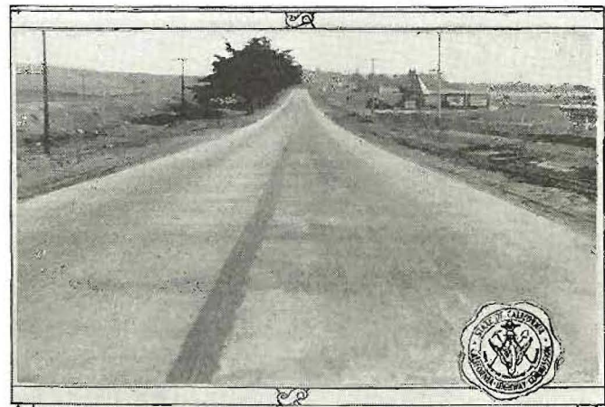
New concrete pavement twenty feet wide with thickened edge and center expansion joint.
