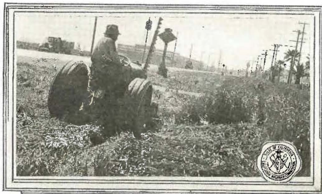
DRESSING UP THE ROADWAY—Mower attachment on a light tractor cutting roadside growth near Stockton. This work improves the appearance of the highway and lessens the fire danger during summer months. (Division X.)
