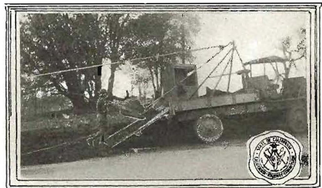
Loading apparatus used by maintenance crew on small shoulder widening jobs. (Division II.)
