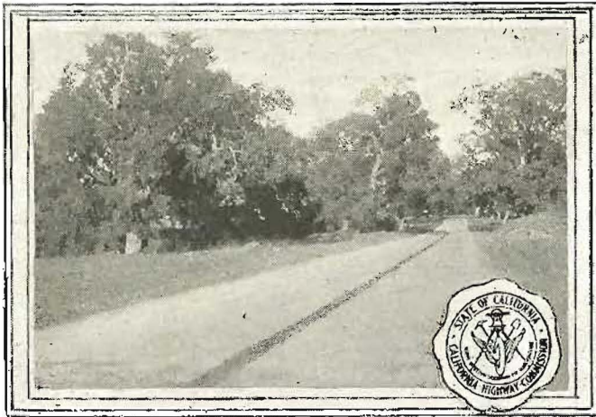
SECOND STORY CONCRETE.—A rebuilt pavement in Ventura County. The new twenty-foot slab was placed over the old fifteen-foot pavement. This was necessary to sustain heavy traffic. (Photo Div. VII.)
