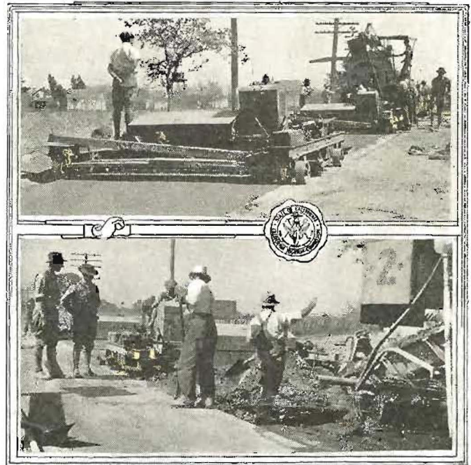
SECOND STORY WORK IN SONOMA.—Placing of new pavement on the Redwood highway, a reconstruction project. Tests show it to be some of the strongest concrete ever placed on the state system. (Photo Div. IV.)
