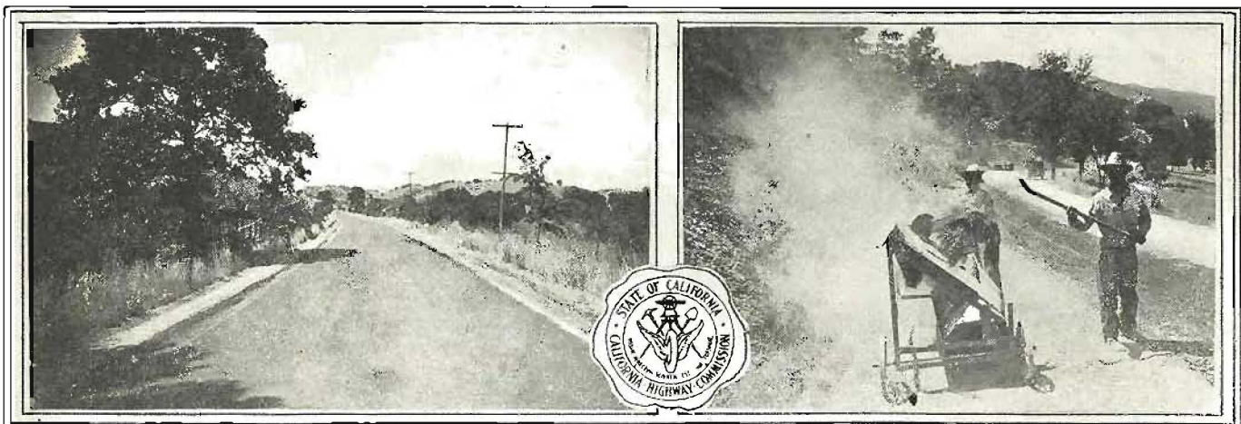
OILING REDWOOD HIGHWAY Experimental oiling of a considerable section of the Redwood highway has been under way during the Summer. Left , newly oiled section of rock-surfaced highway; Right , salvaging rock from the loose material broomed off the highway prior to oiling. Brooming permits oil to penetrate into rock surface. (Photos by Division I.) See article on page, ten.
