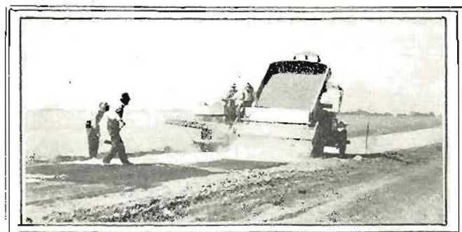
SPREADING ROCK—Division VI outfit on Yosemite lateral where uneven cement pavement was resurfaced with crushed rock and oil. Special spreader arrangement on truck.
