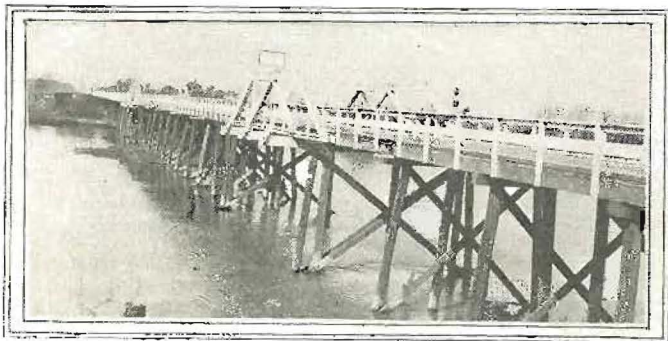
BRIDGE WHICH MUST BE REMOVED—Timber trestle across Sacramento River at Rio Vista which has been ordered replaced by the Federal government by permanent structure to facilitate dredging operations.
