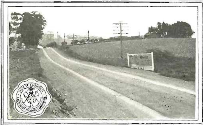
SOUTH OF CARPINTERIA—Division V reconstruction project; cement concrete shoulders and asphalt concrete wearing surface. New width 20 feet
