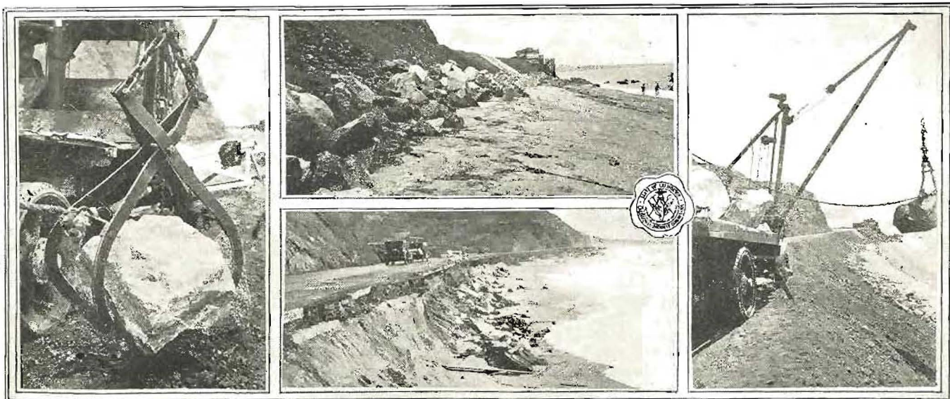
PLACING RIPRAP, DIVISION VII—Trucks equipped with derricks and grappling hooks are in use by maintenance forces of Division VII for placing protection along the coast highway north of Santa Monica. Lower center view shows damage wrought by wave action during storms.
