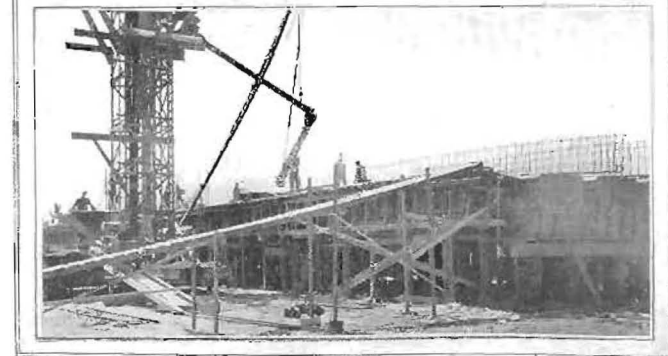
PLANT LAYOUT—Above, central storage and mixing plant on Santa Maria bridge contract; bunkers were filled directly from cars by bucket conveyors; mixer discharged batches directly into reservoir hopper supplying dump car on narrow gauge track. Below, movable hoisting and chuting tower mounted on platform and operating over railroad track; note incline and dump car on hoist platform.
