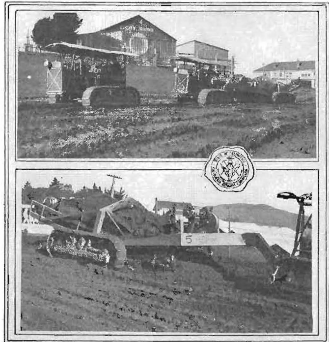
SUPER EARTH MOVER—Views of a Le Tourneau earth mover in use by contractor on Peninsula highway widening project, San Mateo County. Above, caterpillar tractor with snatch; below, mover lifting full load of approximately 15 cubic yards of material.
