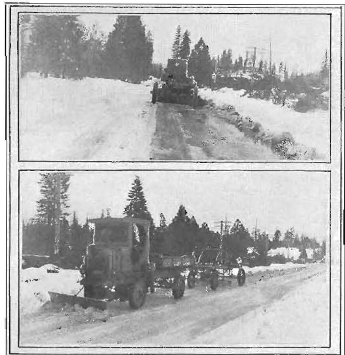
Follow-up crew; maintenance outfit scraping ice from pavement, Pacific highway, after removal of lighter snow by plows. Slippery places are sanded to safeguard traffic.
