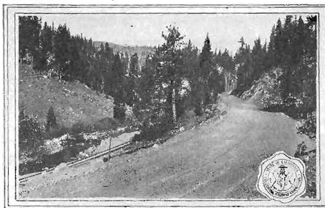
FOREST HIGHWAY—View on new Forest highway under construction by the Bureau of Public Roads between Truckee and Lake Tahoe, in the Tahoe National Forest, Division III. The route is a part of the State highway system.
