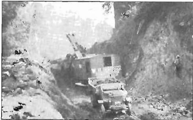
View of heavy excavation being done on Redwood highway contract, north of Orick, Humboldt County.
