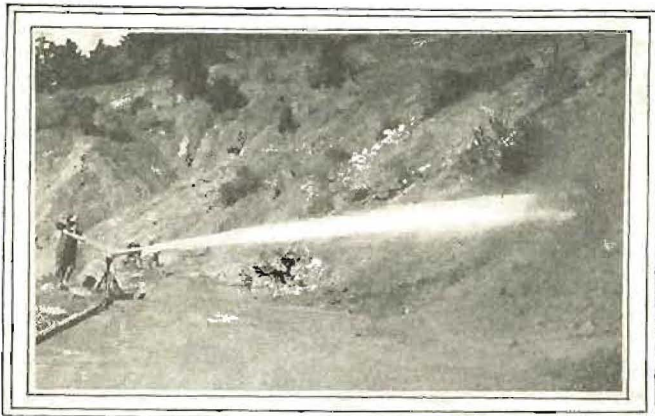
Slide removal by hydraulic jacking on Redwood highway near Garberville, Humboldt County. This method has proved most economical in many locations.
