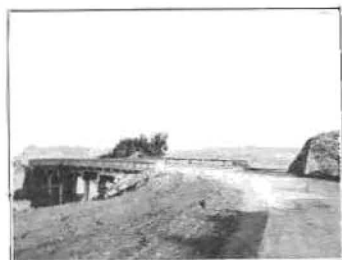
Now we have a separation of grades at the crossing. It is safe for the motorist, and—
