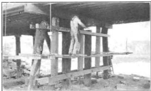
Showing the jacks in place and the crew making the cut-offs. Note the swinging stage from which the men are working.
