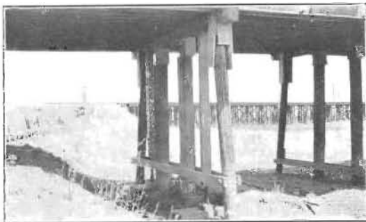
Showing the bents after cut-offs have been made with 4"x12" shims in place and showing part of the scabs holding them in place.
