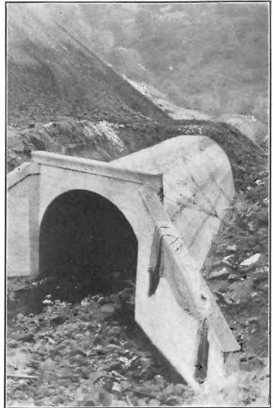
The above concrete culvert was built by men in a prison camp near Oroville, now engaged in building the Feather River lateral to the state highway system.
