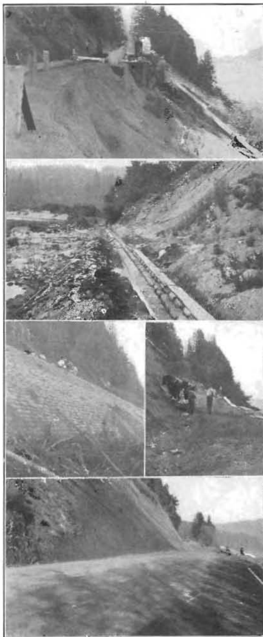
Top view, highway as washed out; middle view, the first tier of sacked cement, view of sacked embankment; filling in back of the sacks; lower view, the widened highway.
