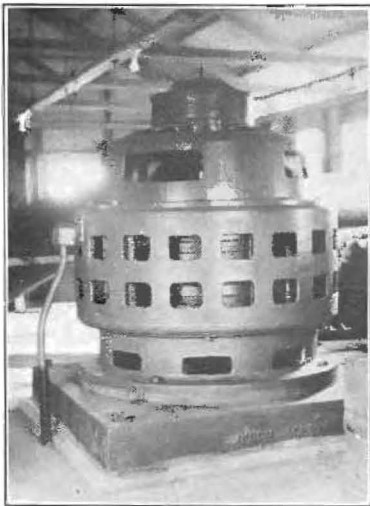
Sutter By-pass, 300-h.p. vertical motor driving a 42-inch pump.
