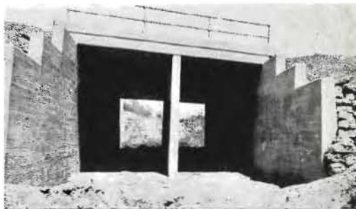
NOW IT STANDS UP , having been rebuilt as a minor improvement without interrupting traffic.
