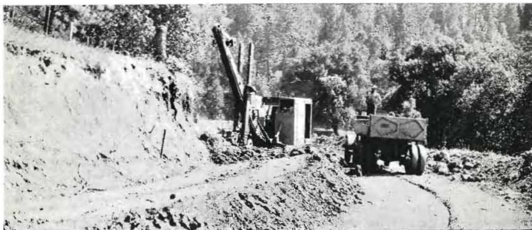
"BLIND BUT DANGEROUS" would have been a fitting warning sign for this curve on the State highway east of Jackson, Amador County, before a rectifying operation classed as a minor improvement corrected it.
