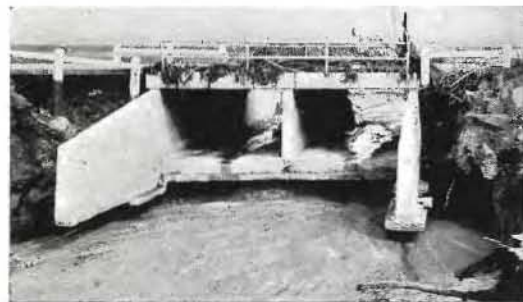
A FLOOD VICTIM , this culvert in Orange County, though widened and deepened, was almost washed out.
