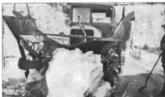
This fixed shovel rotary type machine keeps the road open on the Crest Route near Big Bear Lake, San Bernardino County.
