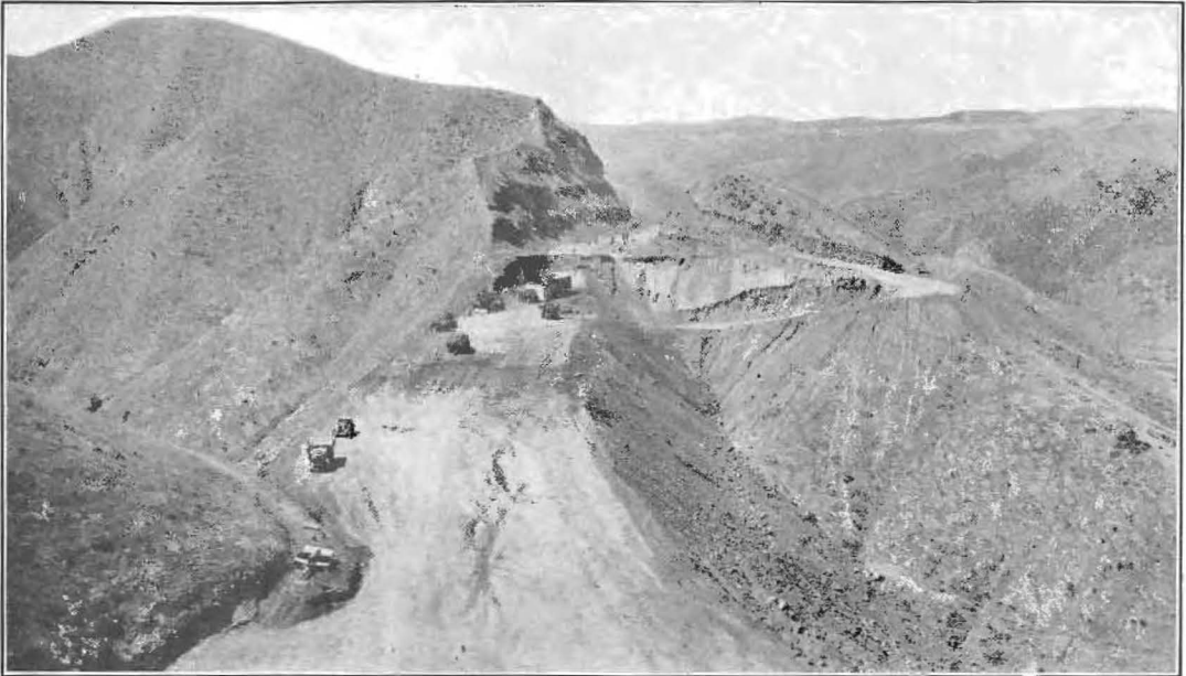
LIKE ANTS ON AN ANT HILL—Putting the finishing touches to a $653,424 highway, the Ridge Route Alternate which will be finished next month. The construction extends over seven miles.
